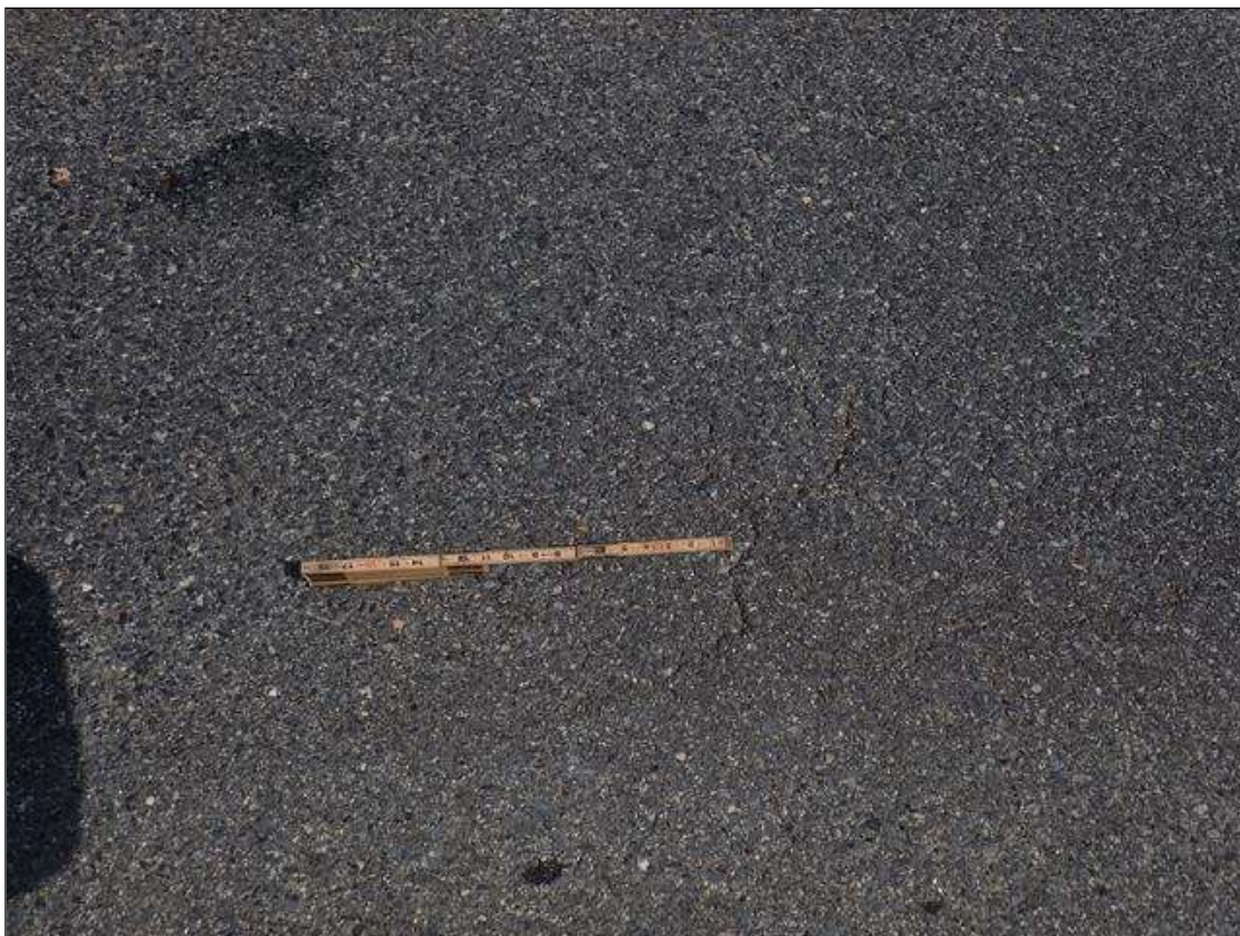
Span 1 Wearing Surface: UP TO 1/16 INCH MAP CRACKING IN VARIOUS LOCATIONS
