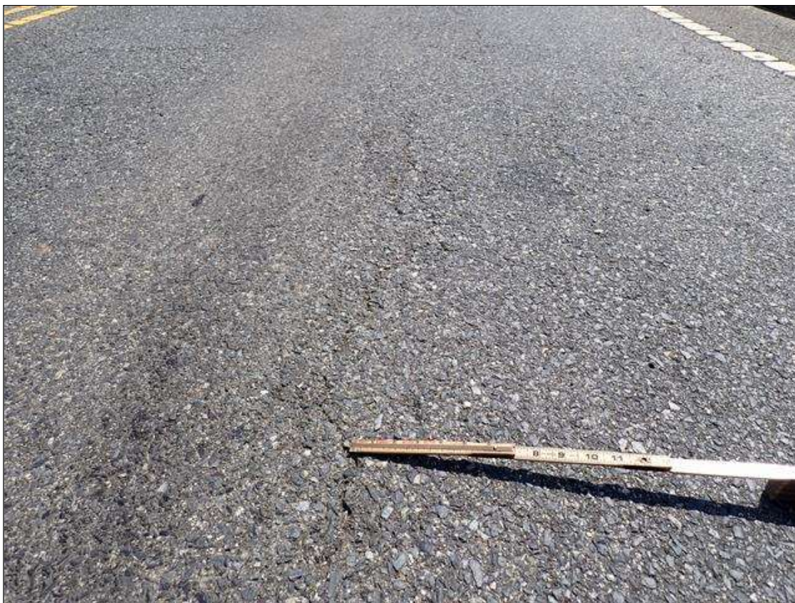
Span 2 Wearing Surface: UP TO 0.016 INCH LONGITUDINAL CRACKS IN VARIOUS LOCATIONS
