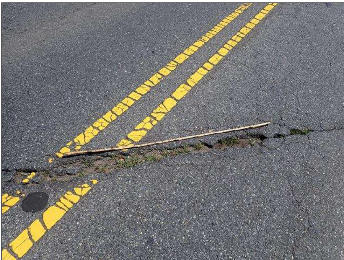
Span 2 Wearing Surface: PAR: UP TO 1/2 INCH WIDE TRANSVERSE CRACKS ALONG BENT 1 WITH (4) SPALLS UP TO 60 INCH X 6 INCH X FULL DEPTH
