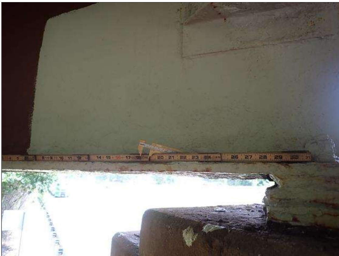
Span 3 Beam 4: PAR: CORROSION ALONG WEB AND BOTTOM FLANGE UP TO 48 INCH LONG X 12 INCH HIGH DOWN TO 7/16 INCH RESIDUAL WEB AND 34 INCH LONG X 12 INCH WIDE DOWN TO 3/8 INCH RESIDUAL BOTTOM FLANGE EXTENDING FROM BENT 2
