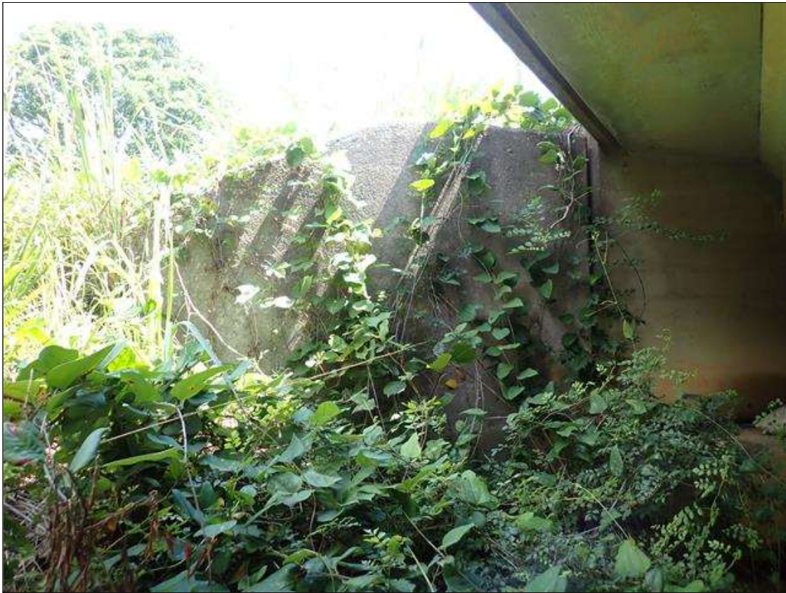
NORTHWEST WINGWALL COVERED IN VEGETATION OVERGROWTH, OTHERS SIMILAR
