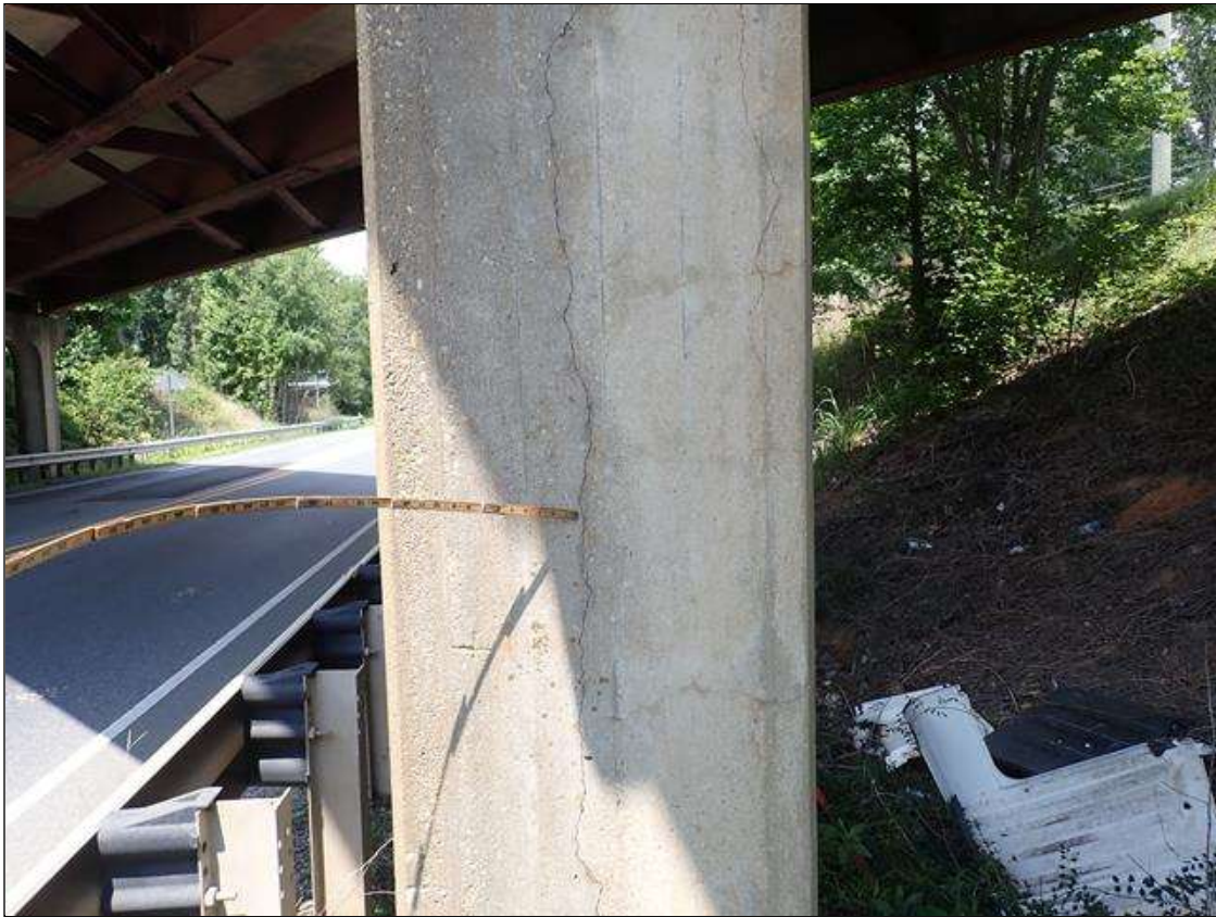
Bent 2 Pile 3: (4) UP TO 9 FEET X 1/16 INCHES VERTICAL CRACKS AT RANDOM THROUGHOUT.
