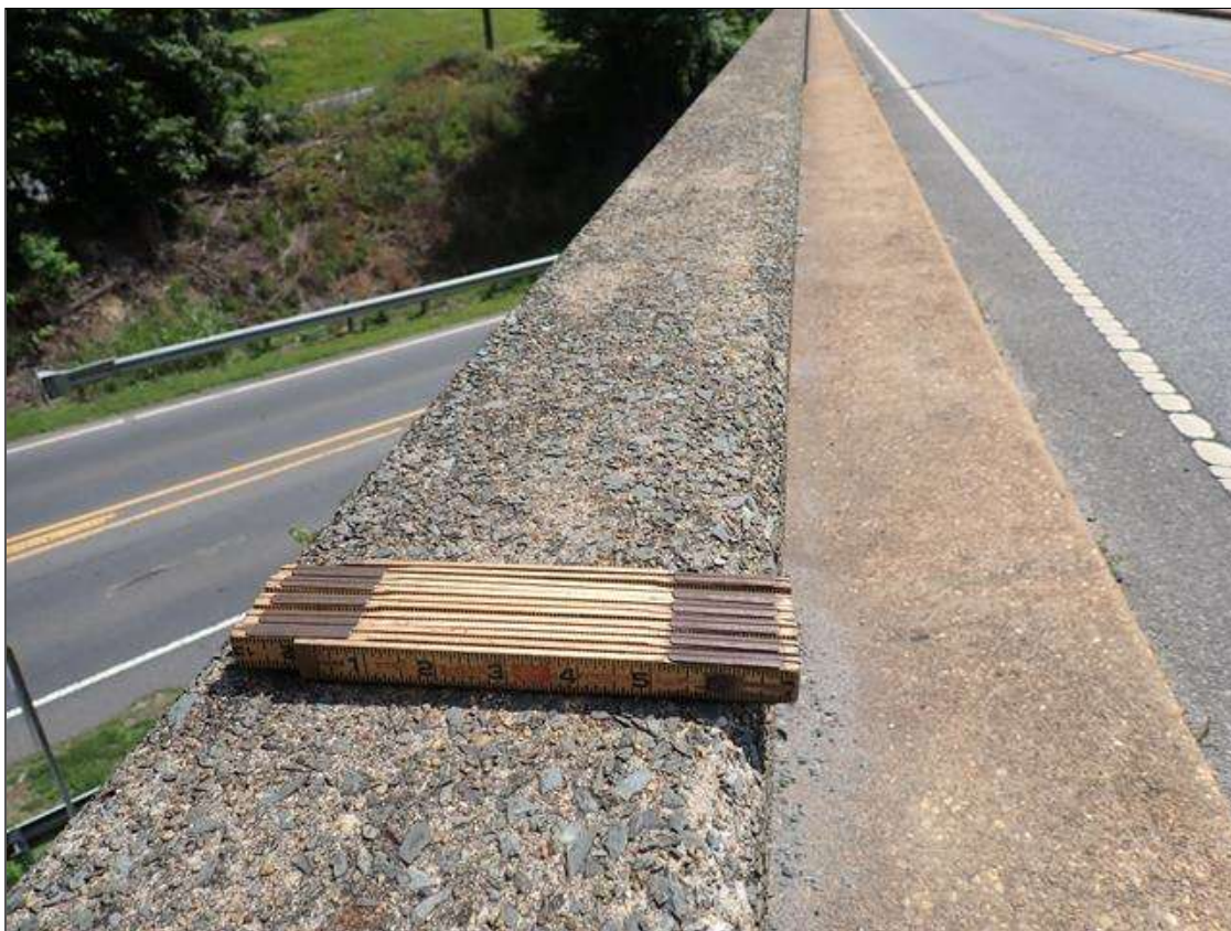
Span 1 Left Bridge Rail: WORN CONCRETE WITH EXPOSED AGGREGATE THROUGHOUT RAIL AND TOP OF CURB
