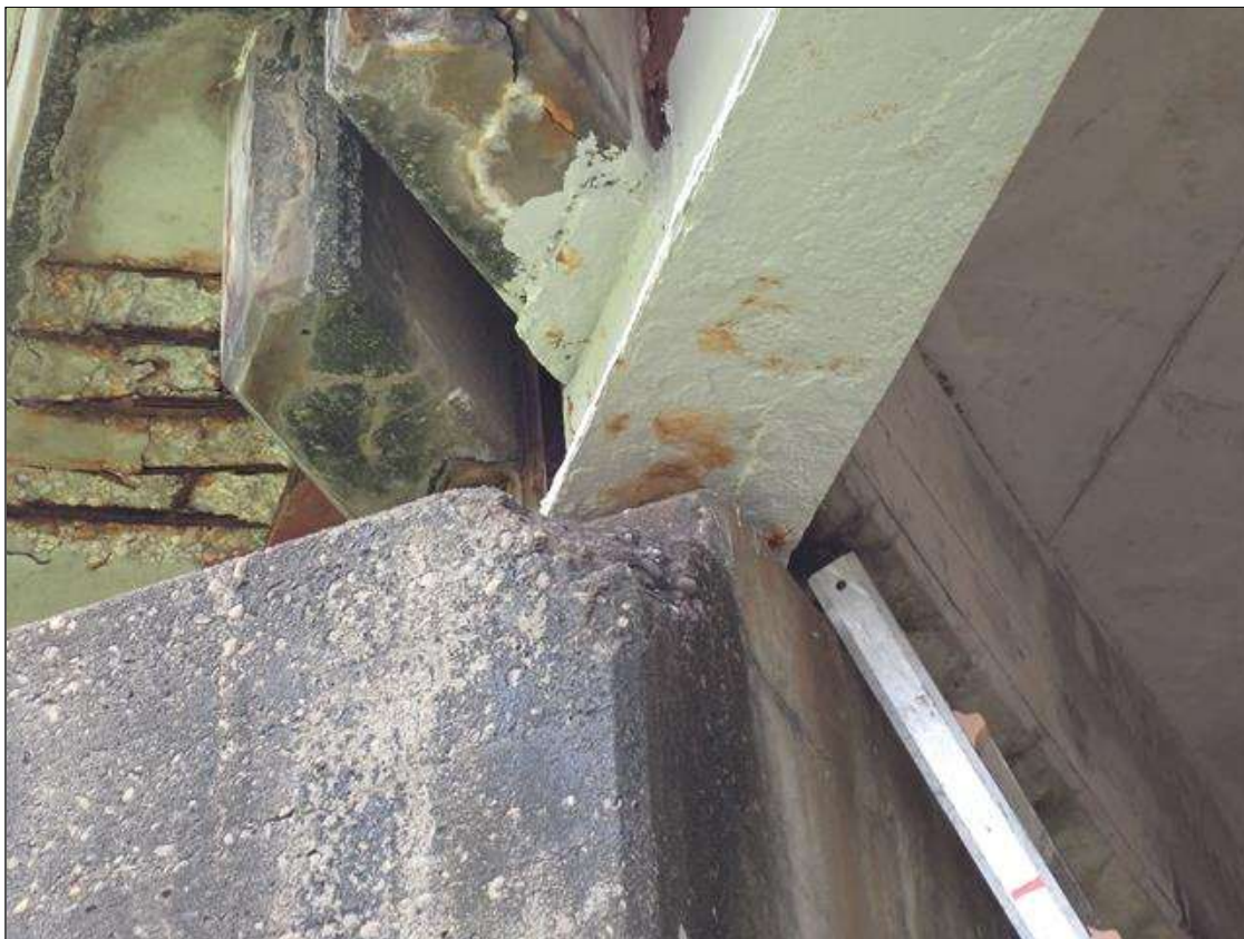
Bent 1 Cap 1: 11 INCHES X 11 INCHES X 5 INCHES SPALL NORTHEAST CORNER.
