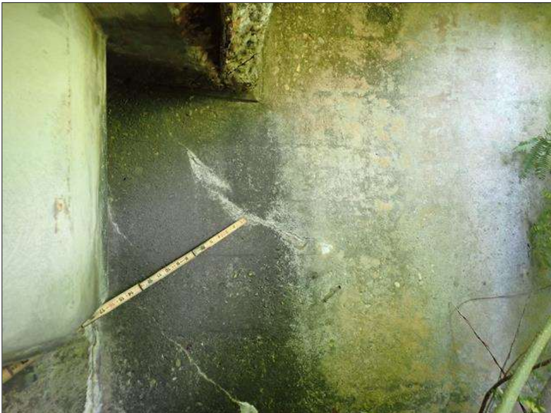
End Bent 1 Abutment: UP TO 0.012 INCH DIAGONAL CRACKS WITH EFFLORESCENCE IN FACE OF BACKWALL BENEATH WEST OVERHANG
