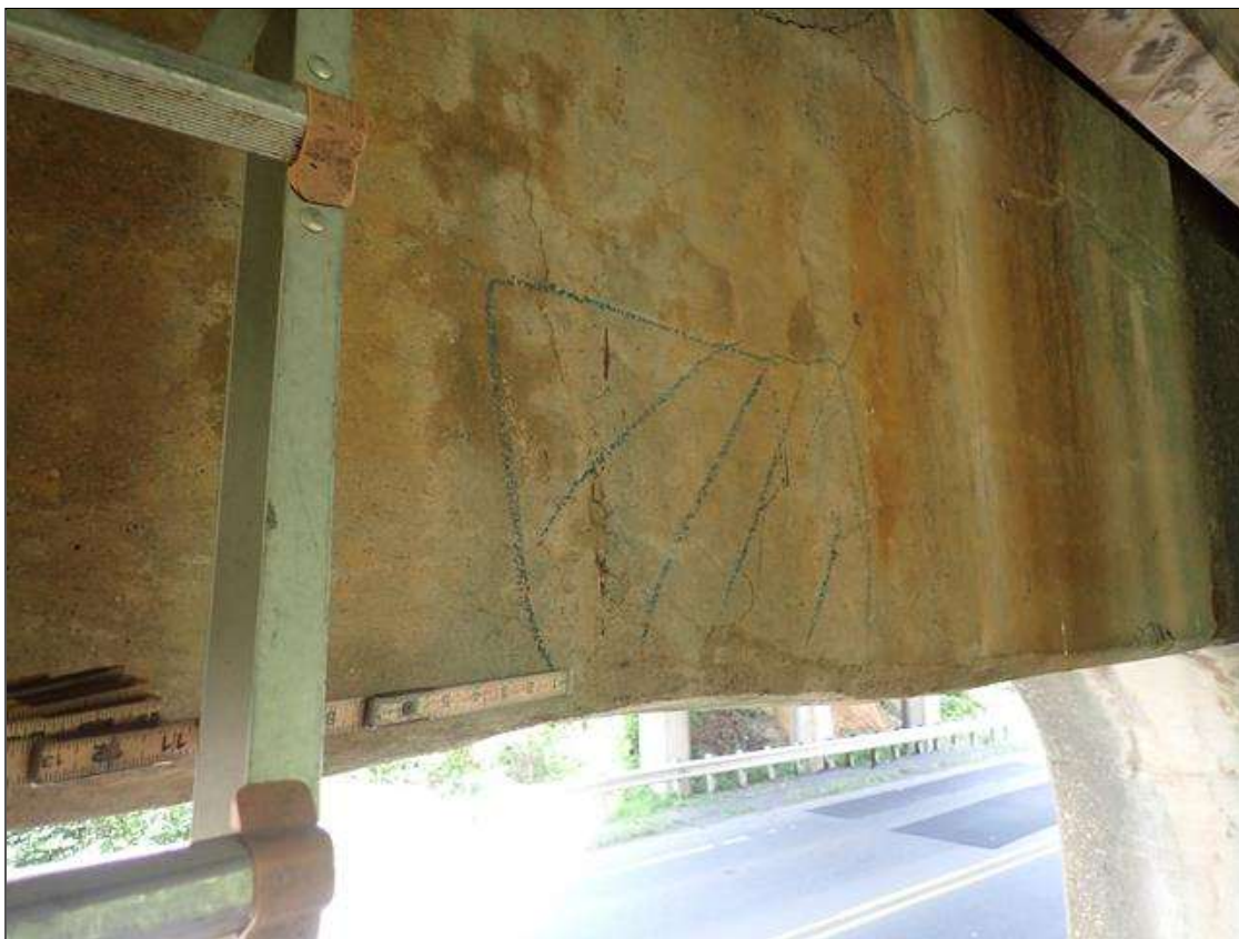
Bent 2 Cap 1: 12 INCHES X 8 INCHES AREA OF DELAMINATION IN NORTH FACE BENEATH BEAM 3.
