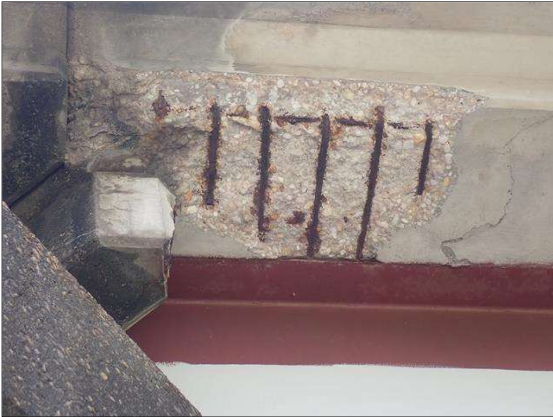
Span 1 Deck: 48 INCH X 30 INCH X 3 INCH SPALL WITH EXPOSED REBAR IN BOTTOM OF DECK IN WEST OVERHANG AT BENT 1.
