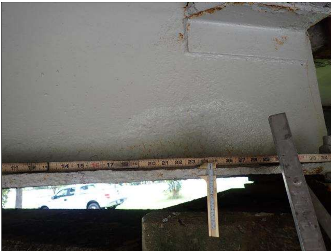
Span 2 Beam 3: PAR: CORROSION ALONG WEB AND BOTTOM FLANGE UP TO 47 INCH LONG X 7 INCH HIGH DOWN TO 3/8 INCH RESIDUAL WEB AND 32 INCH LONG X 12 INCH WIDE DOWN TO 1/2 INCH RESIDUAL BOTTOM FLANGE EXTENDING FROM BENT 1
