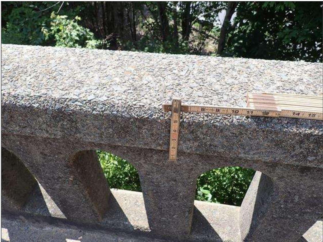
Span 3 Right Bridge Rail: UP TO 0.016 INCH TRANSVERSE AND VERTICAL CRACKS IN TOP AND BOTH FACES OF RAIL IN VARIOUS LOCATIONS
