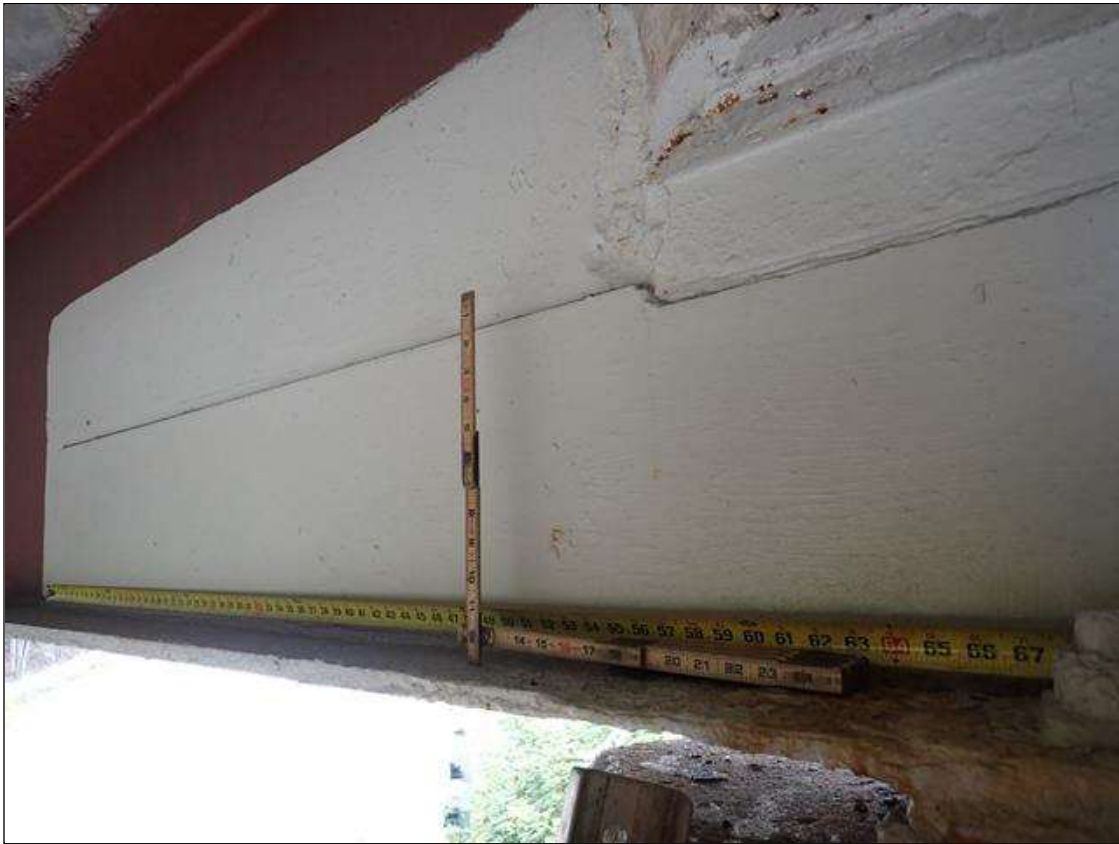
Span 2 Beam 4: 72 INCH X 12 INCH PLATE REPAIR ALONG BOTH FACES OF WEB EXTENDING FROM BENT 1
