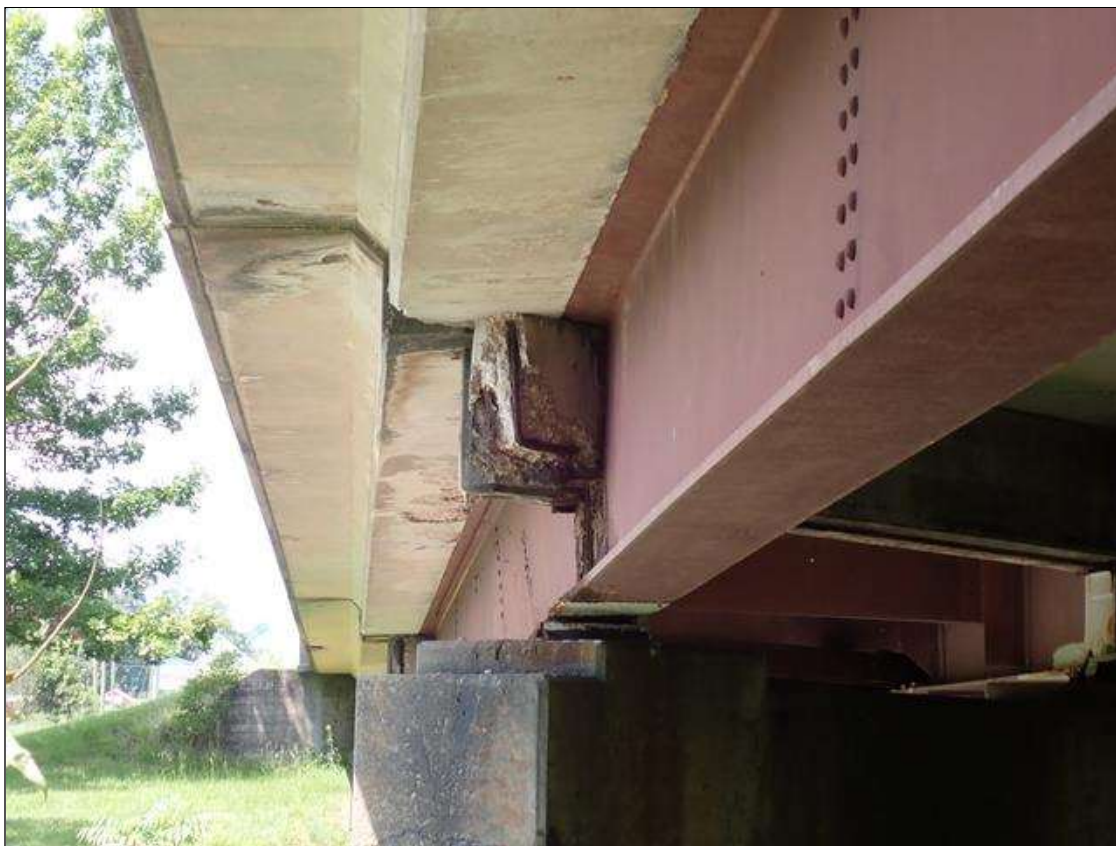
Span 3 Deck: 15 INCHES X 9 INCHES X 4 INCHES DEEP SPALL WITH EXPOSED REBAR AT BENT 2 UNDER EAST OVERHANG.
