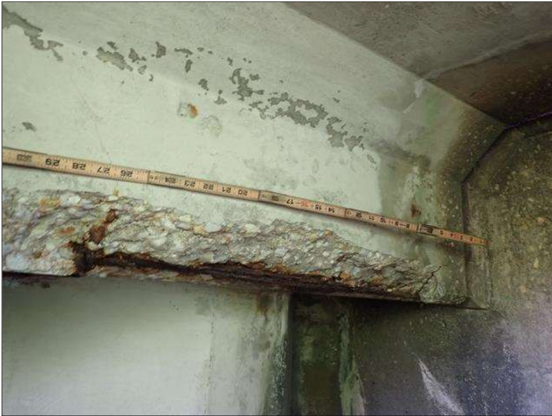
Span 1 Deck: 34 INCH LONG X 7 INCH WIDE X 4 INCH HIGH SPALL WITH EXPOSED REBAR IN BOTTOM AND WEST FACE OF DECK AT END BENT 1
