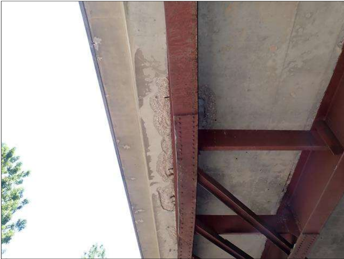
Span 2 Deck: (5) UP TO 48 INCH X 24 INCH X 2 INCHES DEEP SPALLS WITH EXPOSED REBAR IN BOTTOM OF DECK AND EAST OVERHANG ALONG BEAM 3 AND BEAM 4 TOP FLANGE
