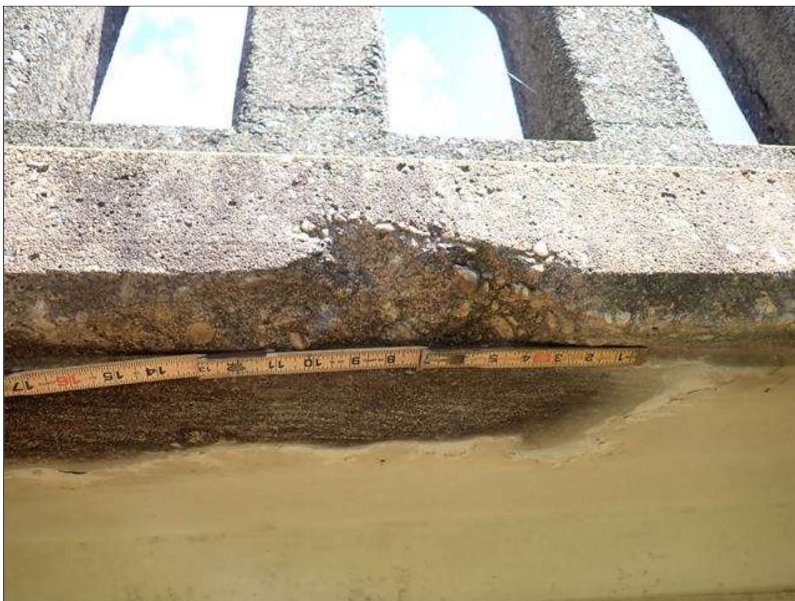
Span 1 Right Bridge Rail: 9 INCHES X 4 INCHES X 2 INCHES DEEP SPALL ON BOTTOM OUTSIDE FACE OF RAIL NEAR MID SPAN
