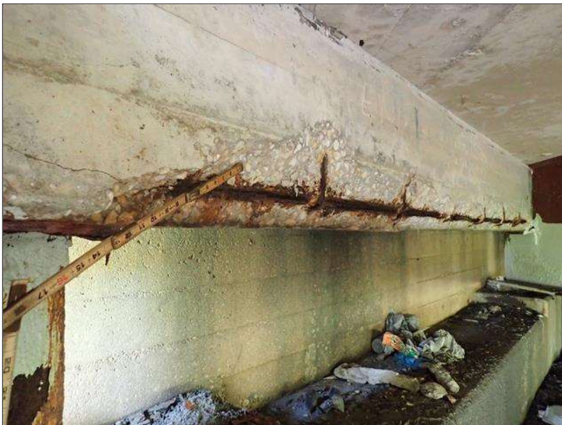
Span 1 Deck: TWO (2) SPALLS WITH EXPOSED REBAR UP TO 11 FOOT LONG X 6 INCH HIGH X 6 INCH WIDE IN END DIAPHRAGMS BETWEEN BEAMS 2 AND 3 AND BEAMS 3 AND 4 AT END BENT 1
