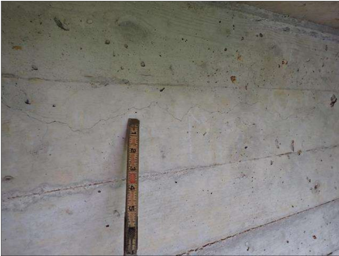
End Bent 2 Abutment: UP TO 0.012 INCH HORIZONTAL CRACKS IN FACE OF BACKWALL IN VARIOUS LOCATIONS
