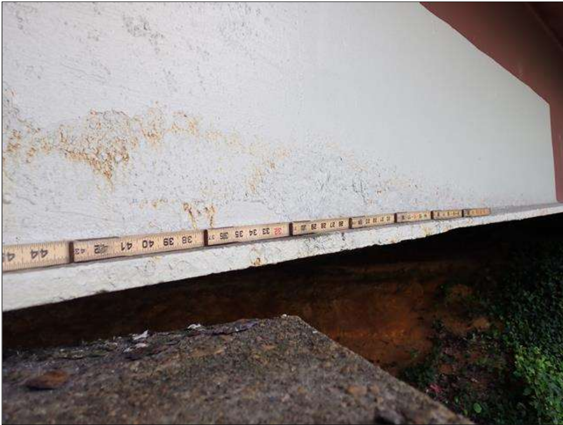
Span 1 Beam 1: PAR: PAINTED OVER AND ARRESTED CORROSION ALONG WEB AND BOTTOM FLANGE UP TO 96 INCH LONG X 8 INCH HIGH DOWN TO 7/16 INCH RESIDUAL WEB AND 96 INCH LONG X 12 INCH WIDE DOWN TO 1/2 INCH RESIDUAL BOTTOM FLANGE, BEGINNING APPROXIMATELY 5 FOOT FROM BENT 1
