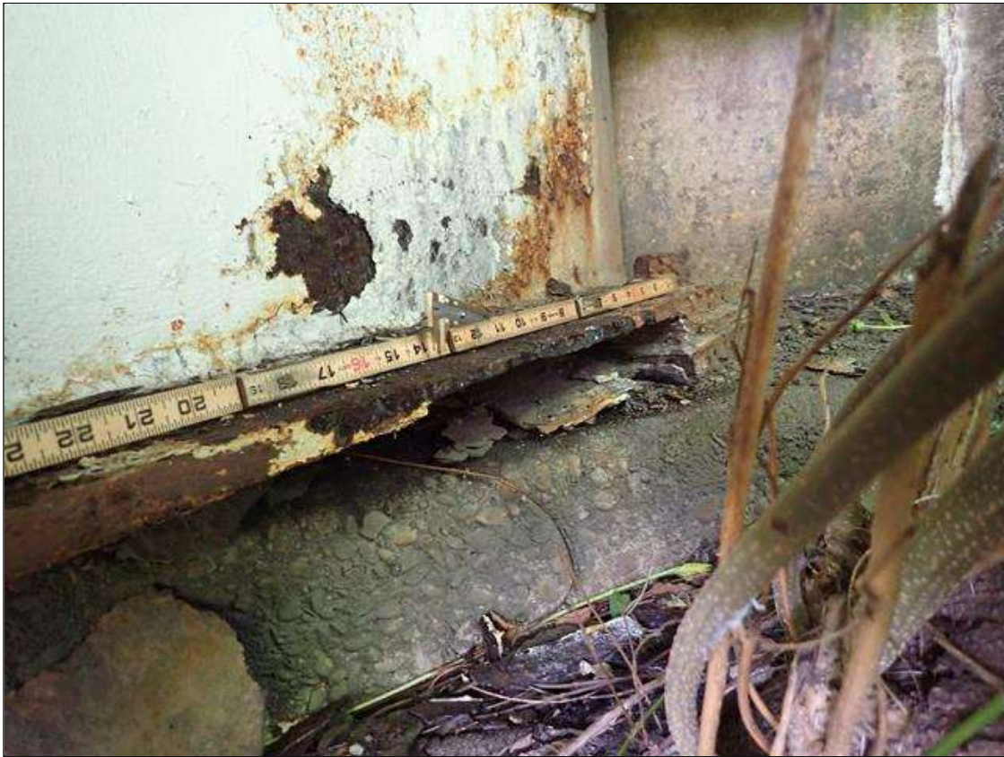
Span 1 Beam 1: PAR: CORROSION ALONG WEB AND BOTTOM FLANGE UP TO 24 INCH LONG X 8 INCH HIGH WITH UP TO 1/16 INCH DEEP PAINTED OVER PITTING IN WEB AND 24 INCH LONG X 6 INCH WIDE DOWN TO 3/8 INCH RESIDUAL BOTTOM FLANGE ON LEFT SIDE EXTENDING FROM END BENT 1
