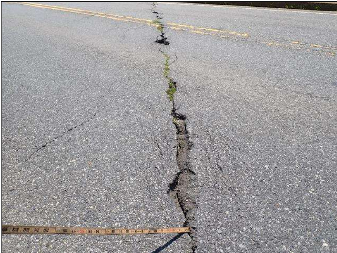
Span 3 Wearing Surface: PAR: UP TO 1/2 INCH WIDE TRANSVERSE CRACKS ALONG END BENT 2 WITH (4) SPALLS UP TO 38 INCH X 5 INCH X FULL DEPTH
