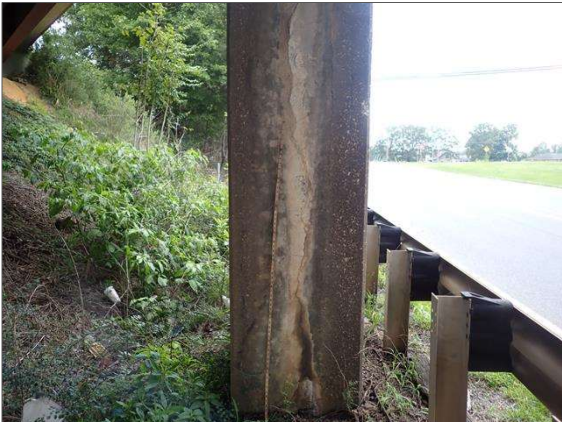
Bent 2 Pile 3: UP TO 0.02 INCH VERTICAL CRACK WITH EFFLORESCENCE BUILD UP AND 96 INCH X 12 INCH AREA OF DELAMINATION IN WEST FACE
