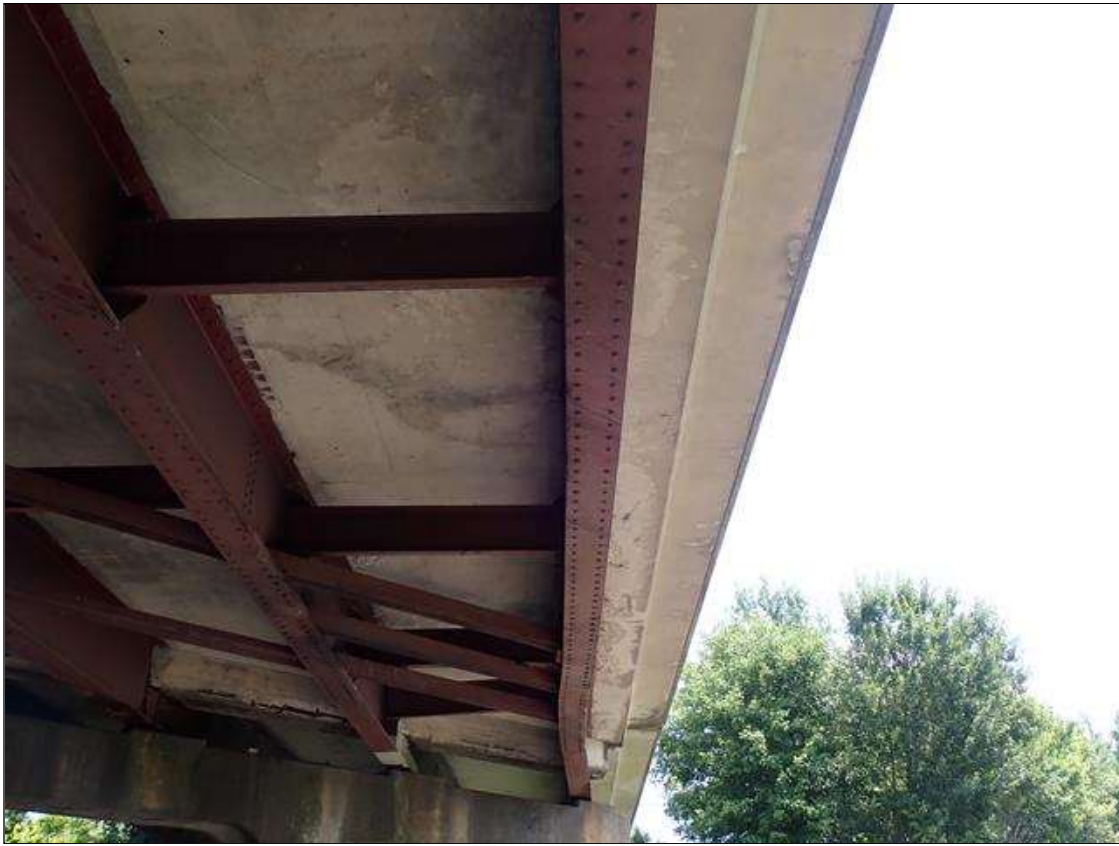
Span 2 Beam 4: IMPACT 9 FEET LONG X UP TO 2 INCHES VERTICAL DISTORTION AND APPROXIMATELY 3 INCHES LATERAL DISTORTION TO BOTTOM FLANGE. NO PAR ISSUED DUE TO LATERAL BRACING ADDED BETWEEN BEAMS PRIOR TO 2021 INSPECTION
