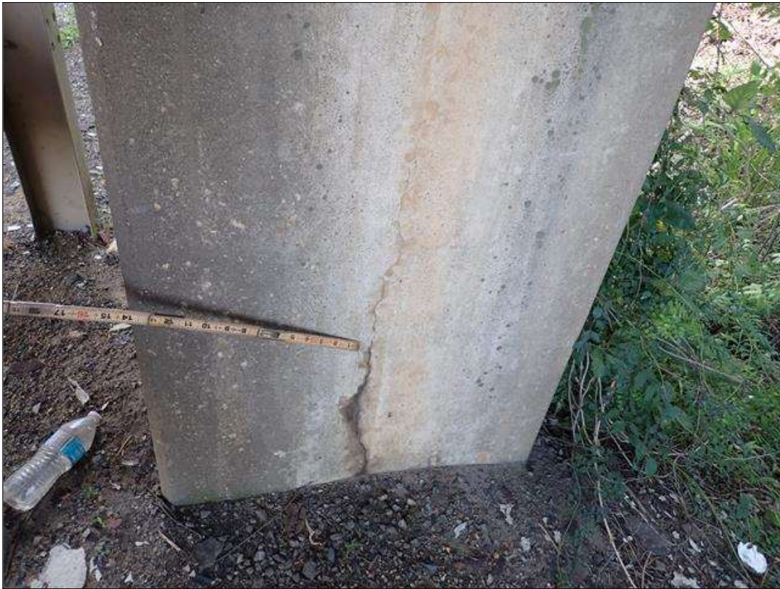
Bent 2 Pile 1: UP TO 0.016 INCH VERTICAL CRACKS IN VARIOUS LOCATIONS
