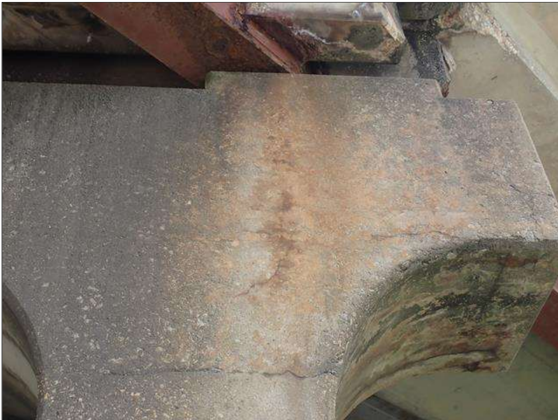
Bent 2 Cap 1: 30 INCH X 30 INCH AREA OF HAIRLINE MAP CRACKING WITH RUST STAINING IN SOUTH FACE AT EAST END.
