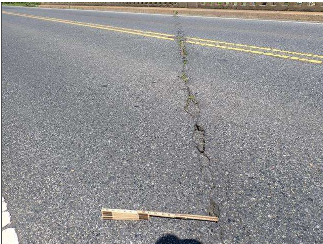
Span 2 Wearing Surface: PAR: UP TO 1/2 INCH WIDE TRANSVERSE CRACKS ALONG BENT 1 WITH (4) SPALLS UP TO 60 INCH X 6 INCH X FULL DEPTH
