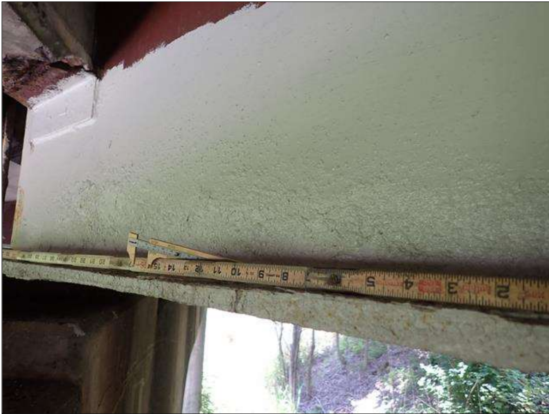
Span 3 Beam 3: PAR: CORROSION ALONG WEB AND BOTTOM FLANGE UP TO 58 INCH LONG X 9 INCH HIGH DOWN TO 7/16 INCH RESIDUAL WEB AND 46 INCH LONG X 12 INCH WIDE DOWN TO 5/8 INCH RESIDUAL BOTTOM FLANGE EXTENDING FROM BENT 2
