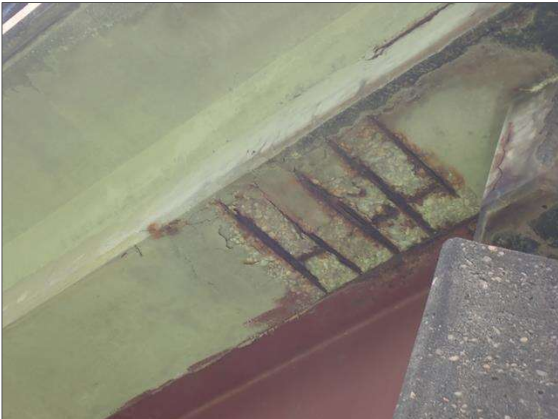
Span 1 Deck: 36 INCH X 30 INCH X 1 INCH DEEP SPALL WITH EXPOSED REBAR IN BOTTOM OF DECK IN EAST OVERHANG AT BENT 1
