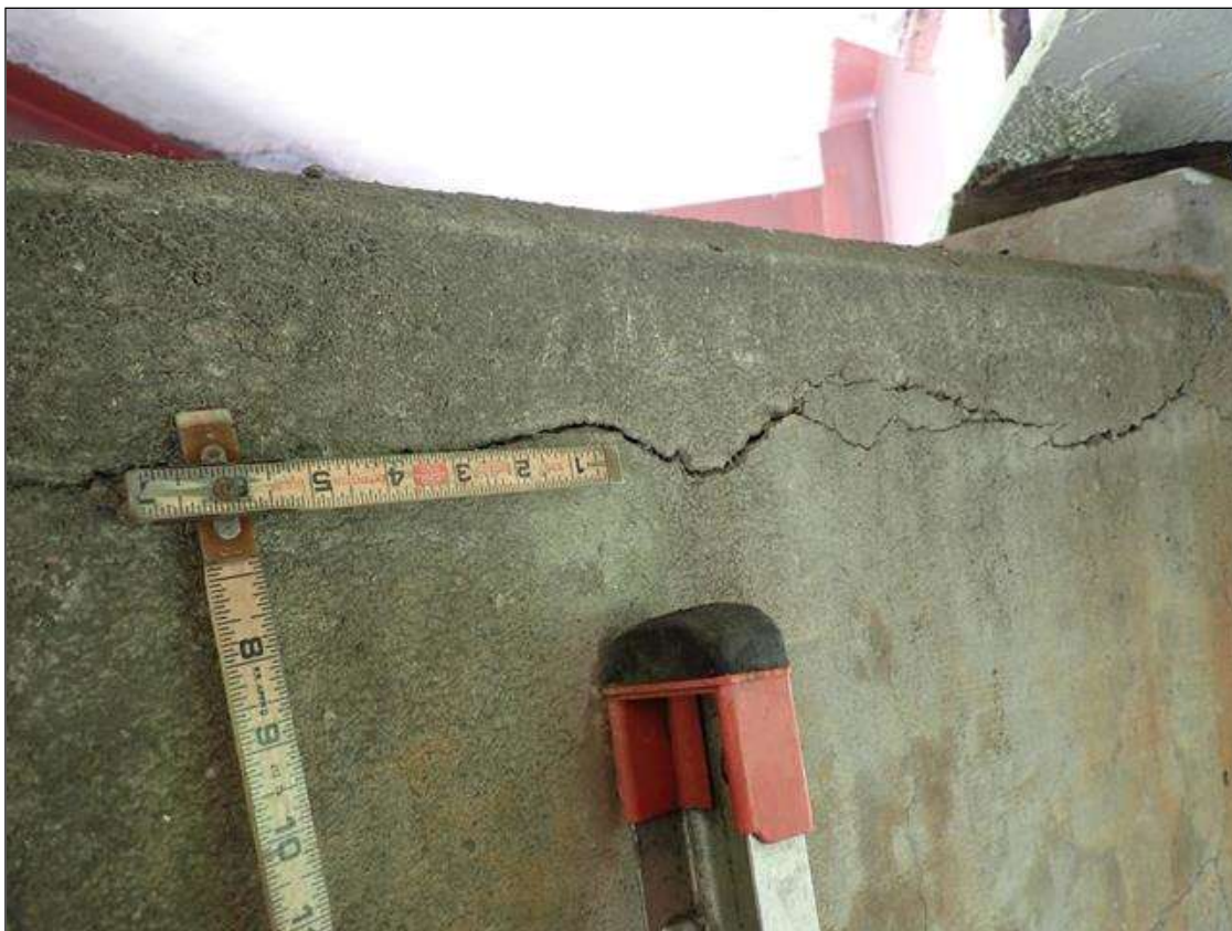
Bent 2 Cap 1: UP TO 1/8 INCH HORIZONTAL CRACKS IN NORTH FACE OF CAP BENEATH BAYS 1 THRU 3
