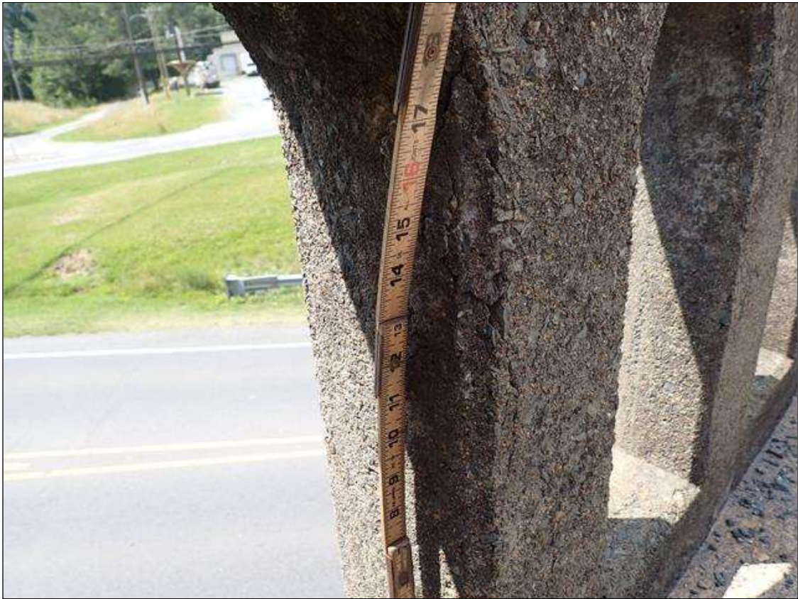
Span 3 Right Bridge Rail: 2 INCHES X 10 INCHES DELAMINATION NORTH FACE RAIL POST 12 FEET FROM BENT 2.
