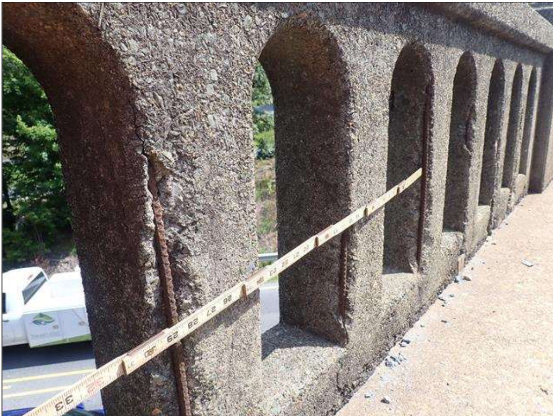
Span 1 Left Bridge Rail: (15) UP TO 3 INCHES X 25 INCHES X 2 INCHES SPALLS WITH EXPOSED REINFORCING AT RANDOM THROUGHOUT RAIL POSTS.
