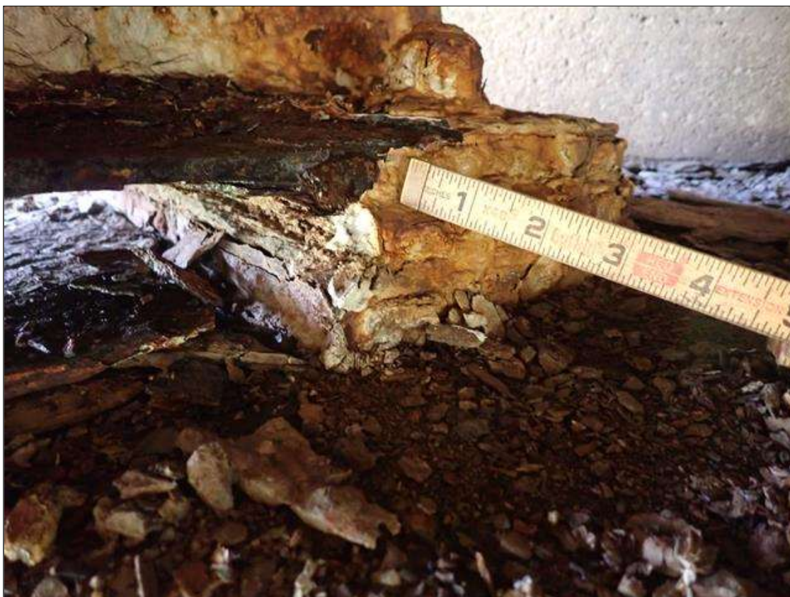
Span 1 Beam 4 - Near Bearing: CORROSION THROUGHOUT
