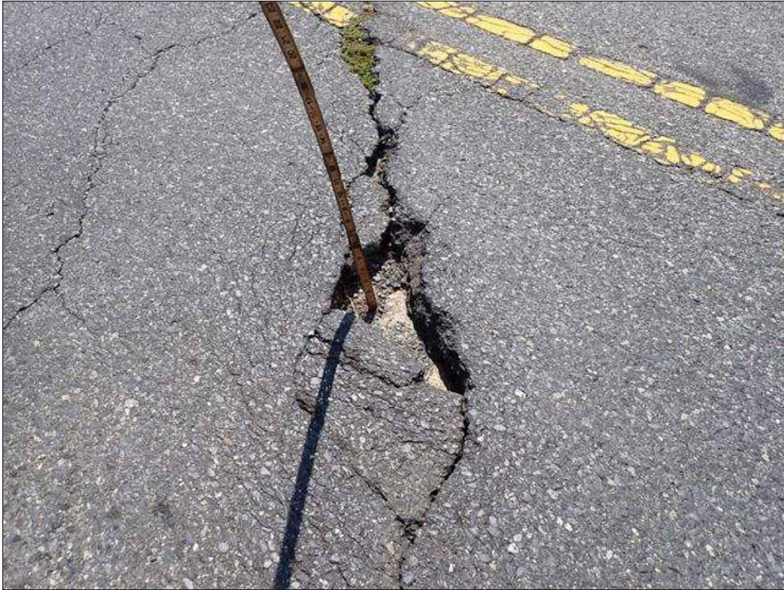
Span 3 Wearing Surface: PAR: UP TO 1/2 INCH WIDE TRANSVERSE CRACKS ALONG END BENT 2 WITH (4) SPALLS UP TO 38 INCH X 5 INCH X FULL DEPTH
