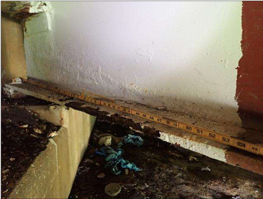
Span 1 Beam 3: PAR: CORROSION ALONG WEB AND BOTTOM FLANGE UP TO 50 INCH LONG X 13 INCH HIGH WITH UP TO 1/16 INCH DEEP PAINTED OVER PITTING IN WEB AND 50 INCH LONG X 6 INCH WIDE DOWN TO 1/2 INCH RESIDUAL BOTTOM FLANGE EXTENDING FROM END BENT 1
