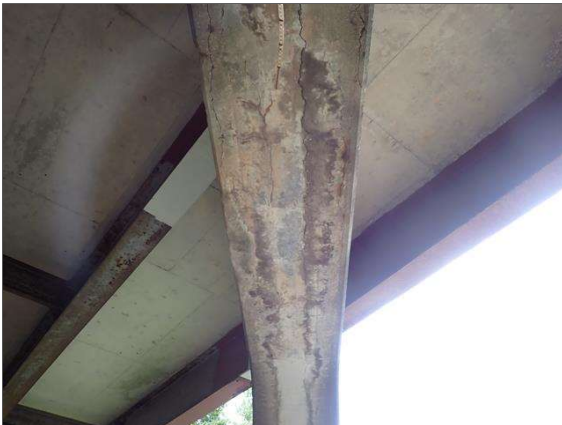
Bent 2 Cap 1: UP TO 1/8 INCH LONGITUDINAL CRACKS AND 13 FOOT LONG X 26 INCH WIDE AREA OF DELAMINATION IN BOTTOM OF CAP BETWEEN COLUMNS 2 AND 3
