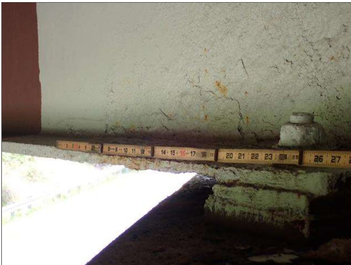
Span 2 Beam 1: PAR: CORROSION ALONG WEB AND BOTTOM FLANGE UP TO 30 INCH LONG X 14 INCH HIGH DOWN TO 3/8 INCH RESIDUAL WEB AND 30 INCH LONG X 12 INCH WIDE DOWN TO 1/2 INCH RESIDUAL BOTTOM FLANGE EXTENDING FROM BENT 2
