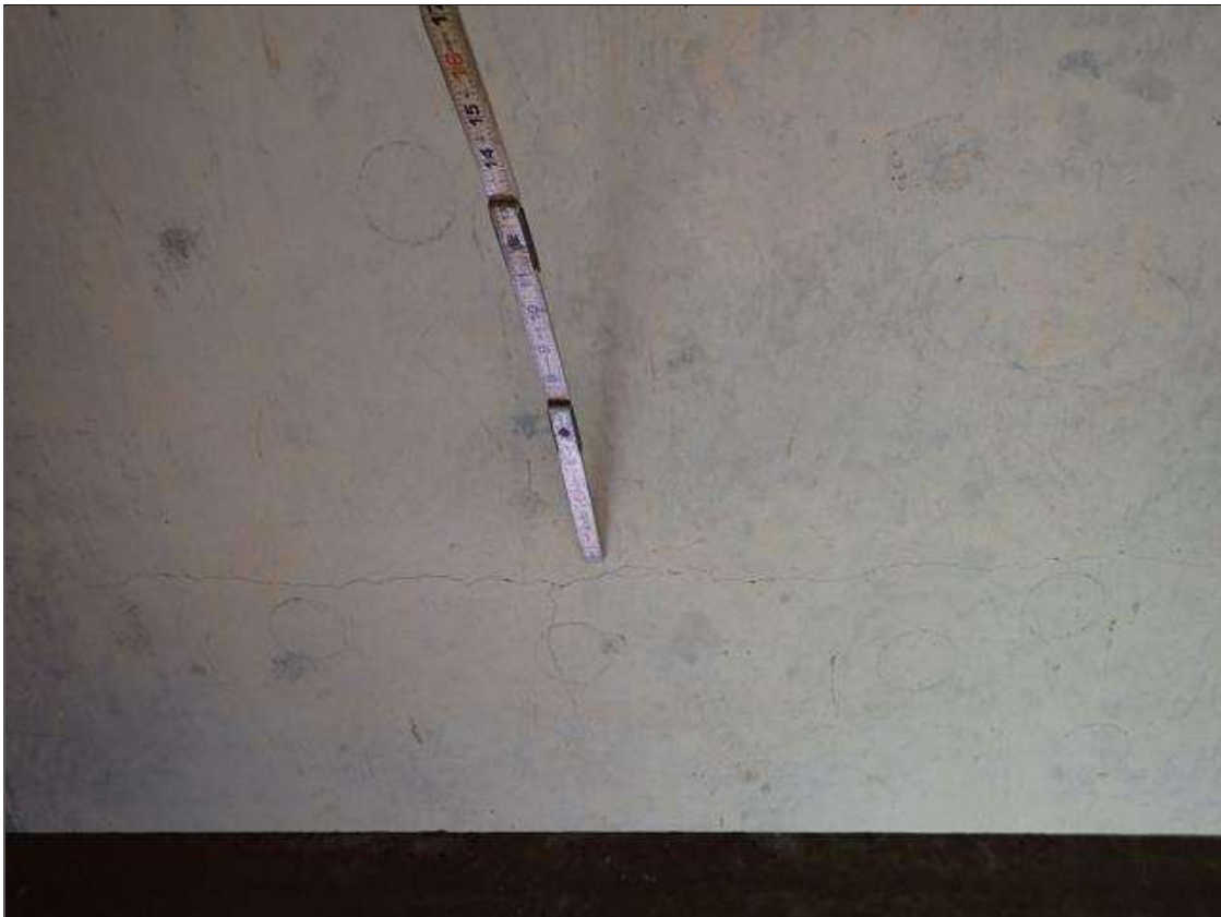
Span 3 Deck: UP TO 0.016 INCH TRANSVERSE CRACKS IN BOTTOM OF DECK IN VARIOUS LOCATIONS
