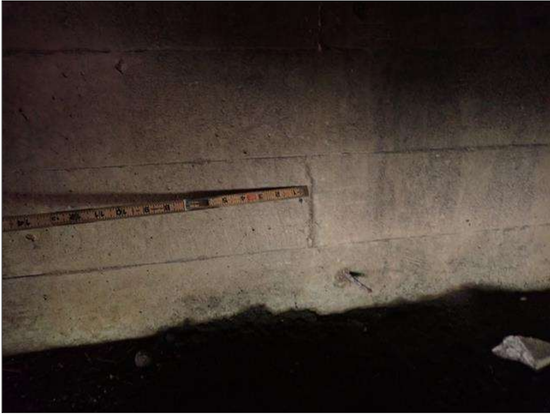
End Bent 1 Abutment: UP TO 1/16 INCH VERTICAL CRACKS IN FACE OF BACKWALL IN VARIOUS LOCATIONS
