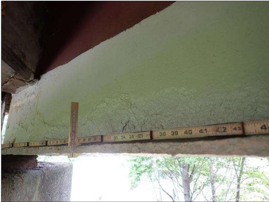
Span 3 Beam 1: PAR: CORROSION ALONG WEB AND BOTTOM FLANGE UP TO 96 INCH LONG X 14 INCH HIGH DOWN TO 3/8 INCH RESIDUAL WEB AND 82 INCH LONG X 12 INCH WIDE DOWN TO 5/8 INCH RESIDUAL BOTTOM FLANGE EXTENDING FROM BENT 2
