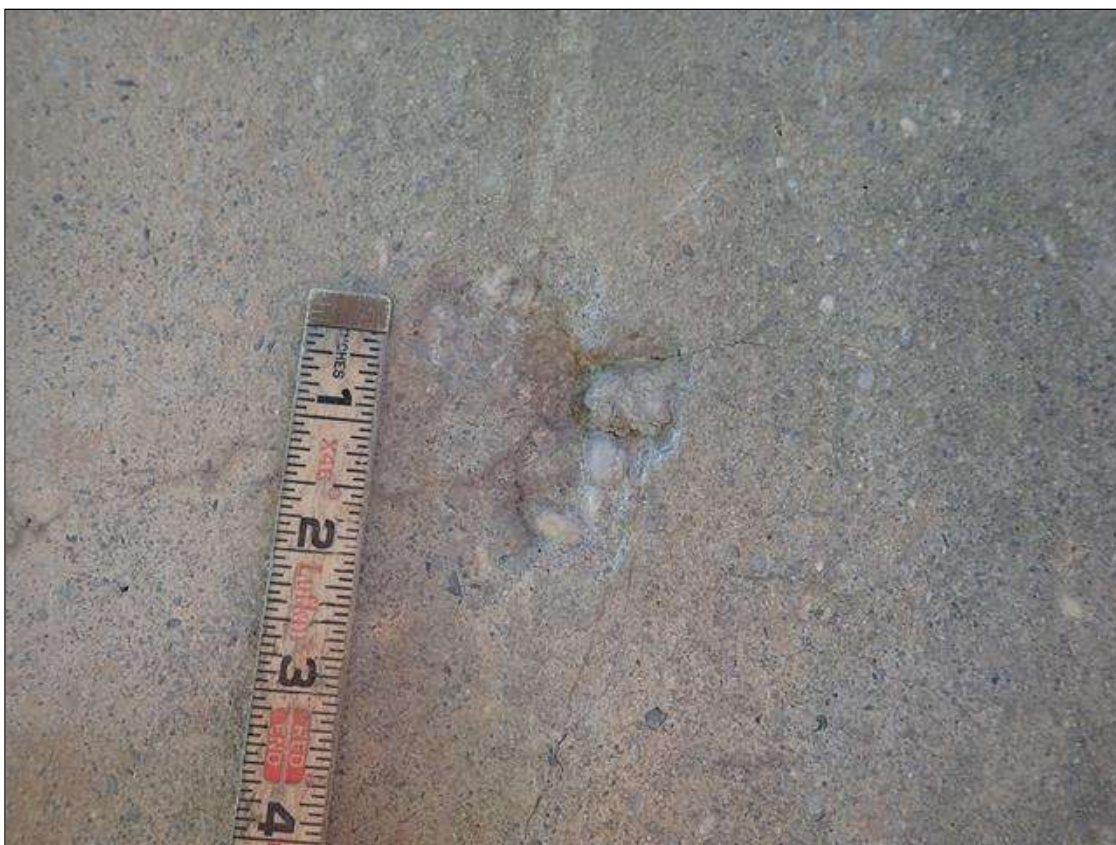
Bent 2 Pile 3: 2 INCHES DIAMETER X 1/2 INCHES DEEP SPALL NORTH FACE 5 FEET FROM BOTTOM OF CAP.
