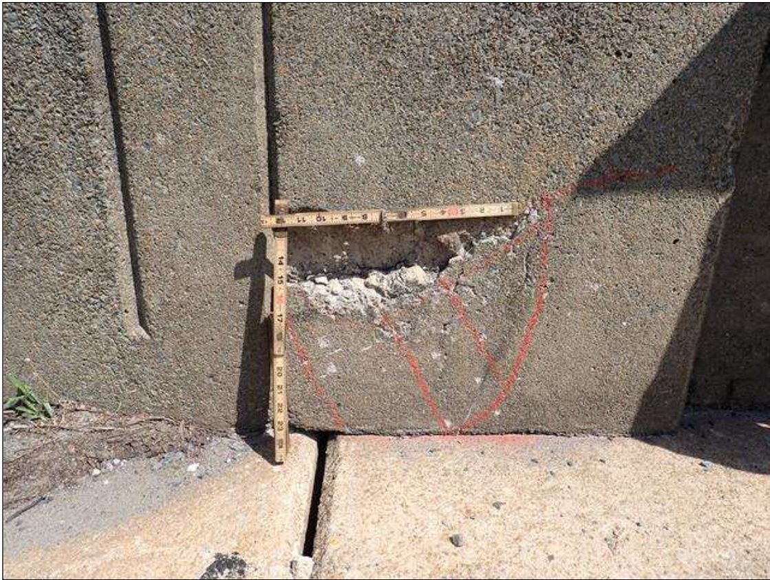
Span 1 Left Bridge Rail: 14 INCH X 12 INCH AREA OF DELAMINATION WITH UP TO 12 INCH X 5 INCH X 2 INCH DEEP SPALL IN FACE OF LEFT RAIL AT END BENT 1
