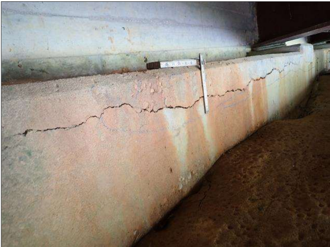
End Bent 2 Cap 1: UP TO 1/4 INCH LONGITUDINAL AND HORIZONTAL CRACKS AND AREA OF DELAMINATION UP TO 20 FOOT LONG X 5 INCH HIGH X 5 INCH WIDE IN TOP AND FACE OF CAP FROM BAY 1 TO BEAM 3
