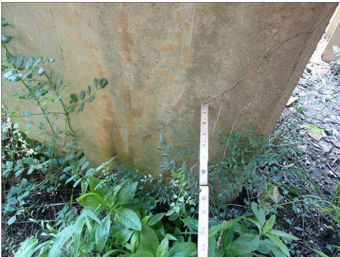
Bent 2 Pile 3: (5) UP TO 1 FEET X 0.016 INCHES DIAGONAL CRACKS AT RANDOM THROUGHOUT NORTH FACE.
