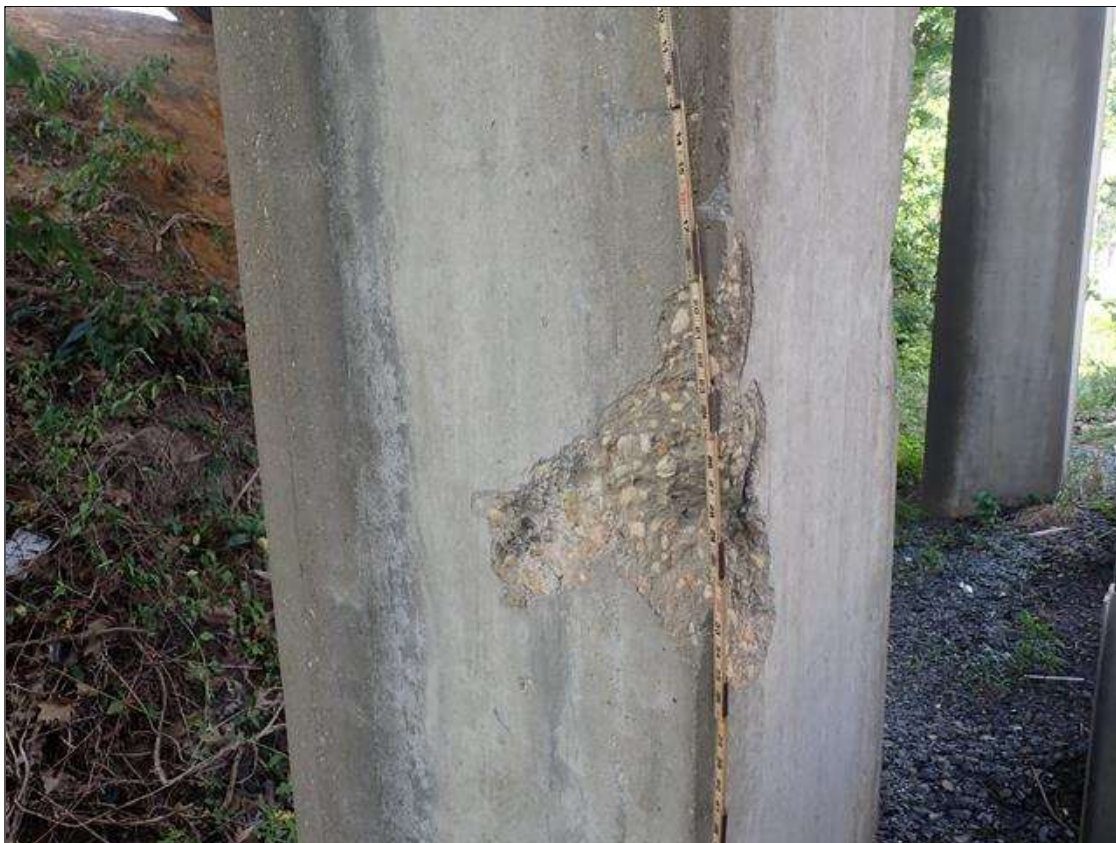
Bent 1 Pile 2: 21 INCHES X 14 INCHES X 6 INCHES SPALL IN NORTHEAST CORNER, APPROXIMATELY 7 FEET FROM BOTTOM OF CAP
