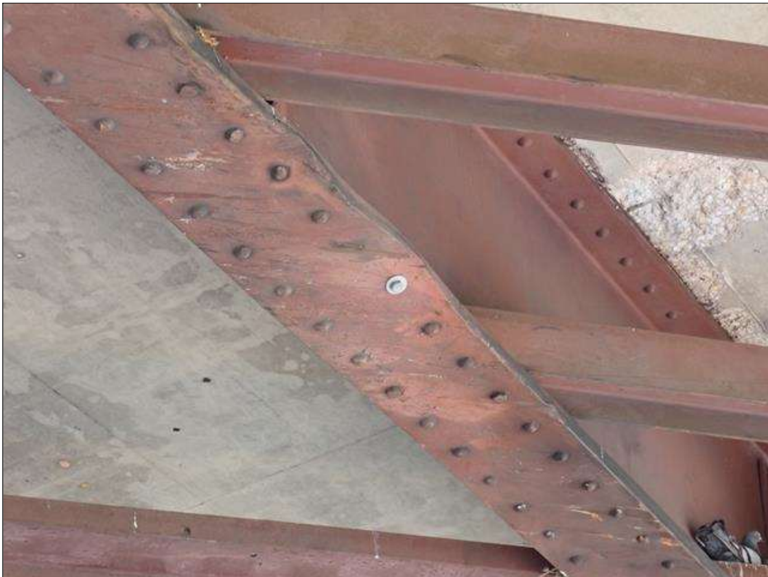
Span 2 Beam 3: MISSING RIVET REPLACED WITH BOLT TO FIX PREVIOUS PAR-- (1) MISSING BOLT IN COVER PLATE CONNECTION 19 FEET FROM BENT 2. PRIOR TO 2021 INSPECTION
