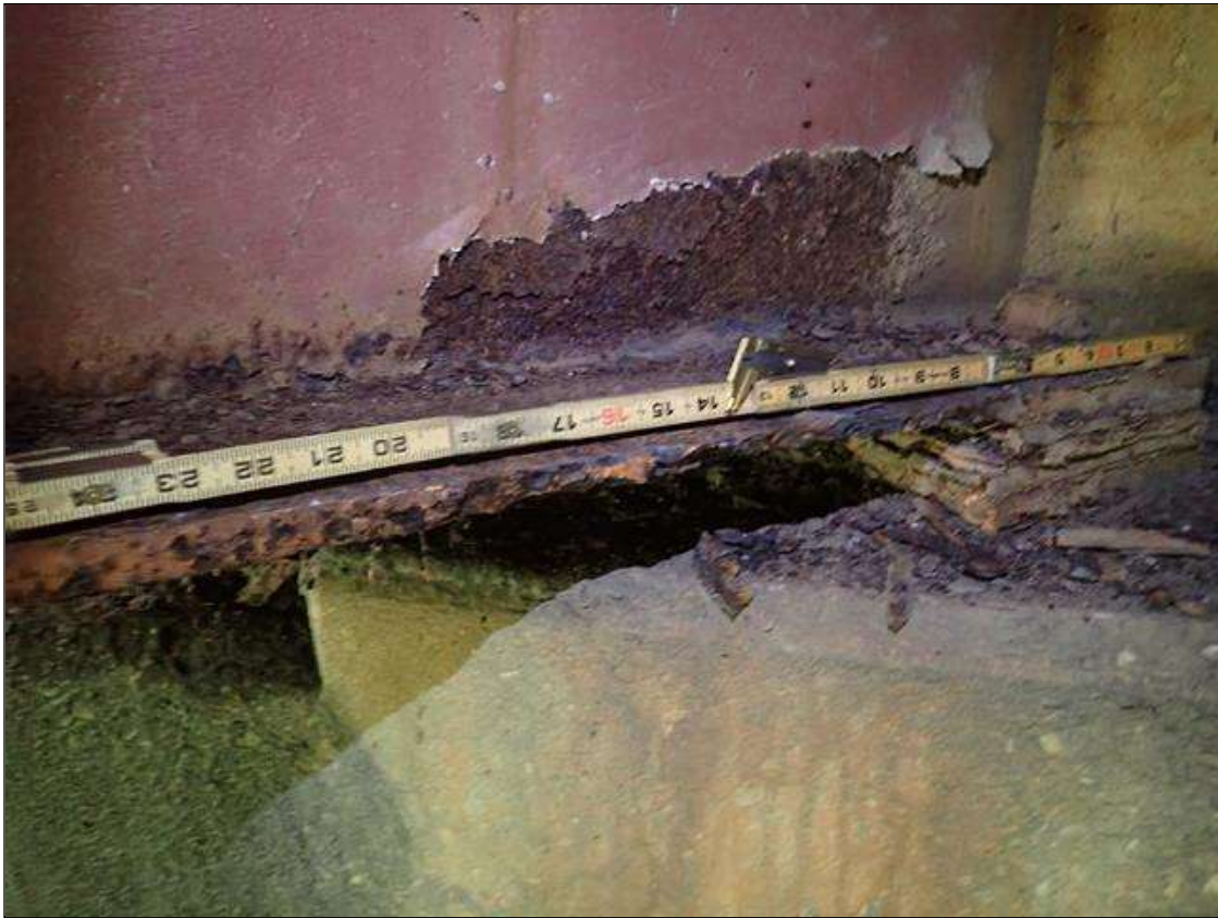
Span 1 Beam 2: PAR: CORROSION ALONG WEB AND BOTTOM FLANGE UP TO 46 INCH LONG X 5 INCH HIGH WITH NO MEASURABLE LOSS OF SECTION IN WEB AND 46 INCH LONG X 6 INCH WIDE DOWN TO 3/8 INCH RESIDUAL BOTTOM FLANGE EXTENDING FROM END BENT 1
