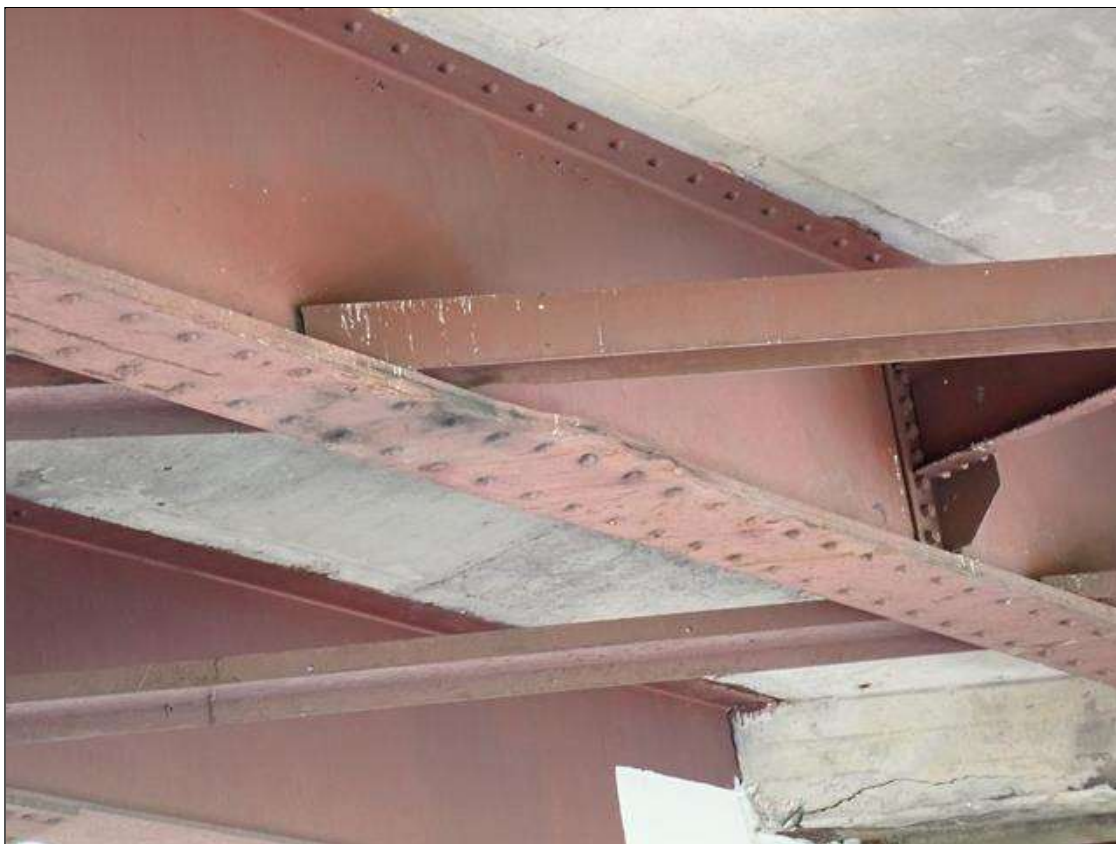
Span 2 Beam 2: 30 INCH LONG X UP TO 1.5 INCHES DISTORTION TO BOTTOM FLANGE 19.5 FEET FROM BENT 2.
