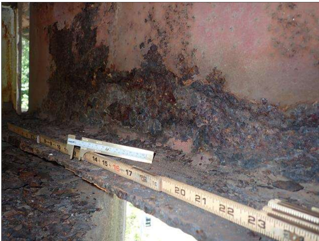
Span 2 Beam 1: PAR: CORROSION ALONG WEB AND BOTTOM FLANGE UP TO 69 INCH LONG X 12 INCH HIGH DOWN TO 1/4 INCH RESIDUAL WEB AND 69 INCH LONG X 12 INCH WIDE DOWN TO 3/8 INCH RESIDUAL BOTTOM FLANGE EXTENDING FROM BENT 1
