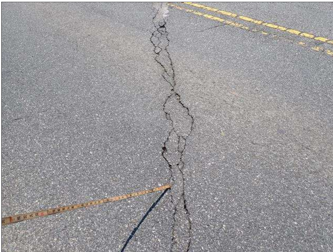
Span 3 Wearing Surface: UP TO 1/2 INCH TRANSVERSE CRACKS AND 96 INCH X 8 INCH AREA OF ALLIGATOR CRACKS ALONG BENT 2
