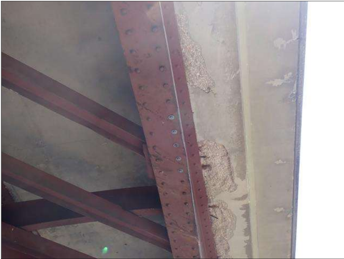
Span 2 Beam 4: RIVETS HAVE BEEN REPLACED WITH BOLTS TO REPAIR PREVIOUS PAR-- (5) MISSING BOLTS IN COVER PLATE CONNECTION AT MID SPAN. PRIOR TO 2021 INSPECTION
