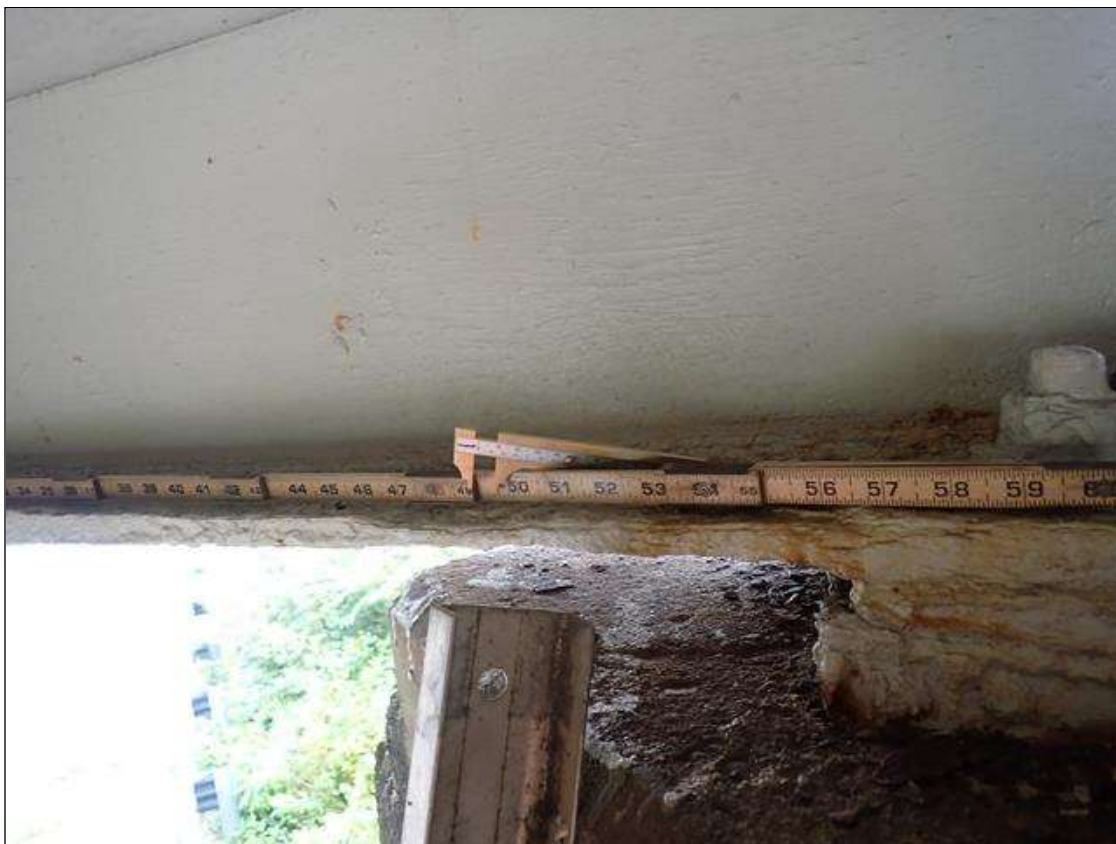
Span 2 Beam 4: PAR: CORROSION ALONG BOTTOM FLANGE UP TO 72 INCH LONG X 12 INCH WIDE DOWN TO 1/2 INCH RESIDUAL BOTTOM FLANGE EXTENDING FROM BENT 1
