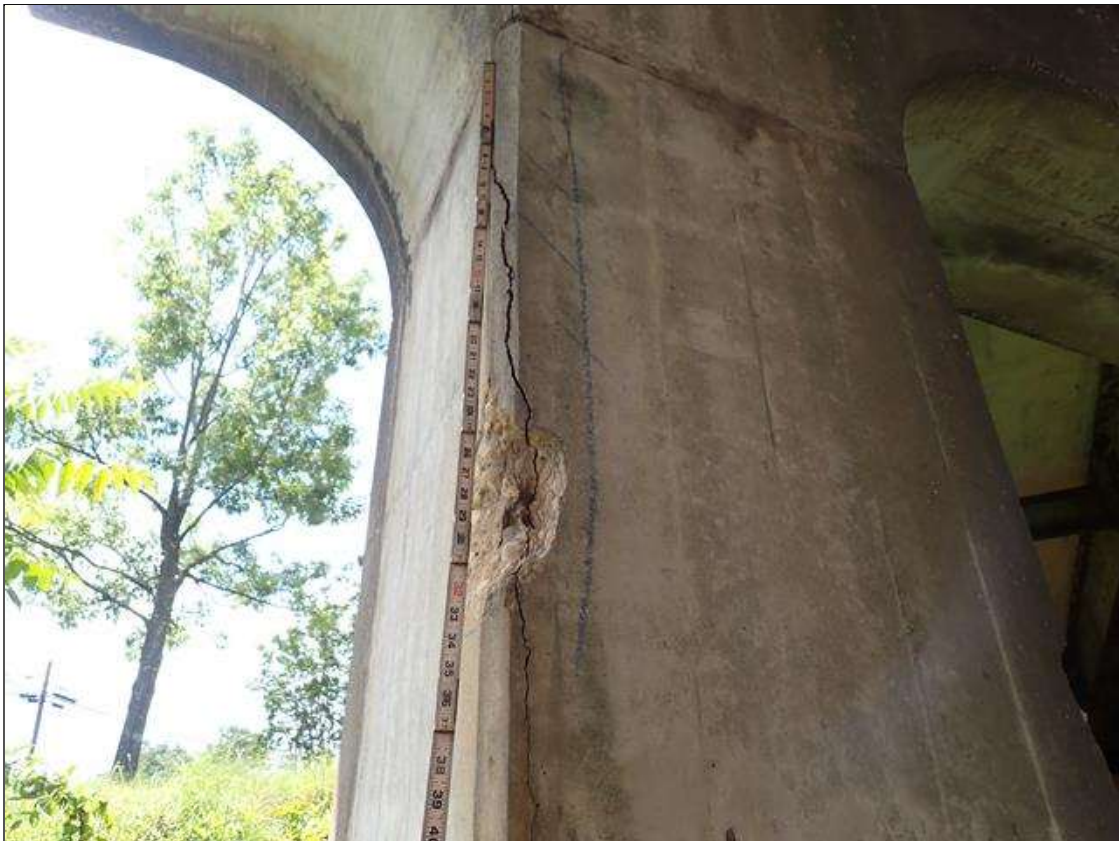
Bent 1 Pile 3: (2) UP TO 10 INCHES X 7 INCHES X 2 INCHES SPALLS WITH UP TO 24 INCHES X 4 INCHES AREA OF DELAMINATION ALONG NORTH CORNERS
