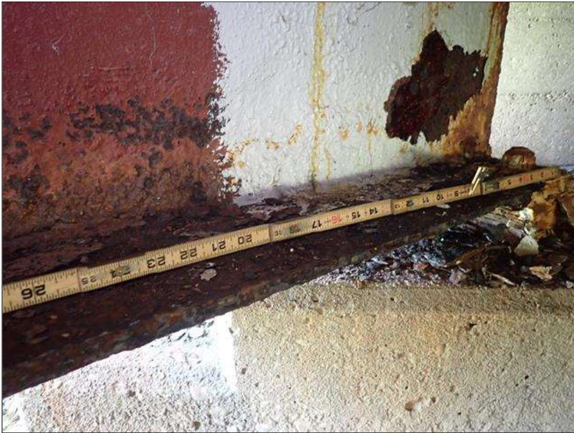
Span 1 Beam 4: PAR: CORROSION ALONG WEB AND BOTTOM FLANGE UP TO 58 INCH LONG X 12 INCH HIGH DOWN TO 3/8 INCH RESIDUAL WEB AND 58 INCH LONG X 6 INCH WIDE DOWN TO 5/16 INCH RESIDUAL BOTTOM FLANGE EXTENDING FROM END BENT 1
