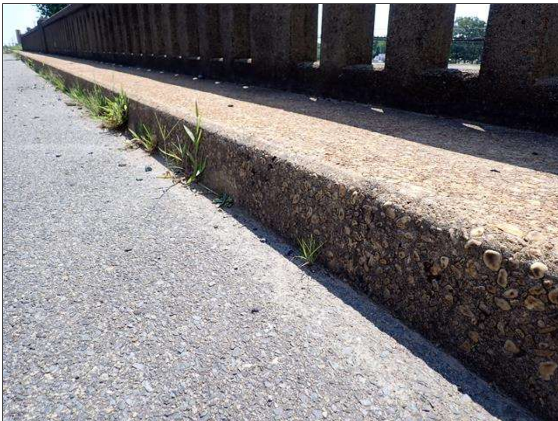
DIRT AND DEBRIS ACCUMULATION WITH VEGETATION GROWTH ALONG BOTH SHOULDERS
