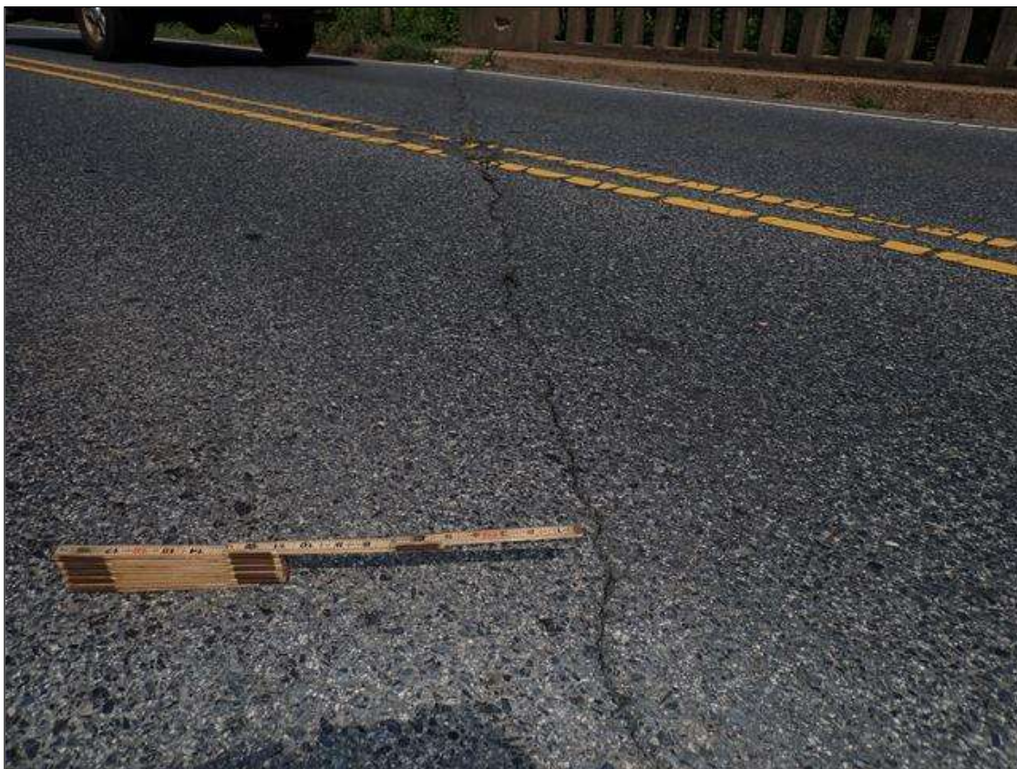
Span 1 Wearing Surface: UP TO 3/4 INCH WIDE TRANSVERSE CRACK ALONG END BENT 1 FILL FACE
