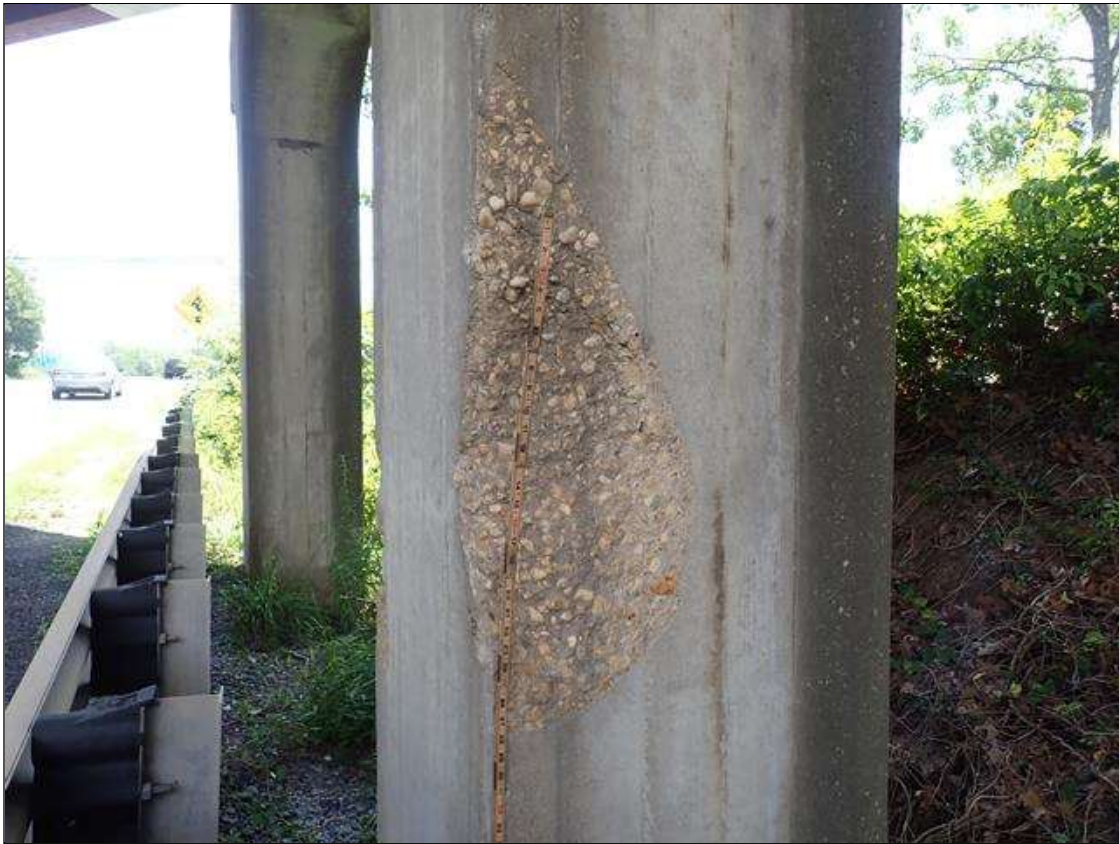
Bent 1 Pile 2: 35 INCH X 15 INCH X 4 INCH SPALL IN NORTHWEST CORNER OF PILE, APPROXIMATELY 6 FOOT FROM BOTTOM OF CAP
