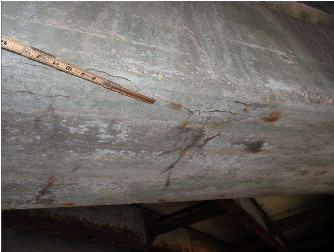
Bent 1 Cap 1: 6 FEET X 12 INCHES DELAMINATION BOTTOM OF CAP BETWEEN PILES 1 AND 2.
