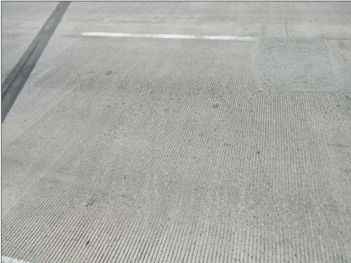
Span 3 Wearing Surface: LATEX MODIFIED CONCRETE WEARING SURFACE HAS SCATTERED MAP CRACKS.
