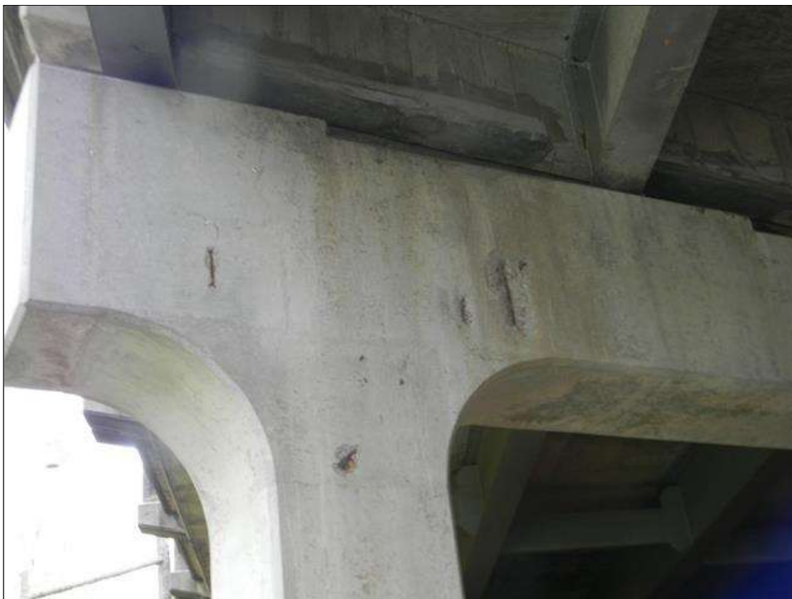
Bent 2 Cap 1: WEST FACE OF CAP UNDER BAY 1 HAS 3 AREAS OF EXPOSED REBAR (4", 3", 10" LONG).
