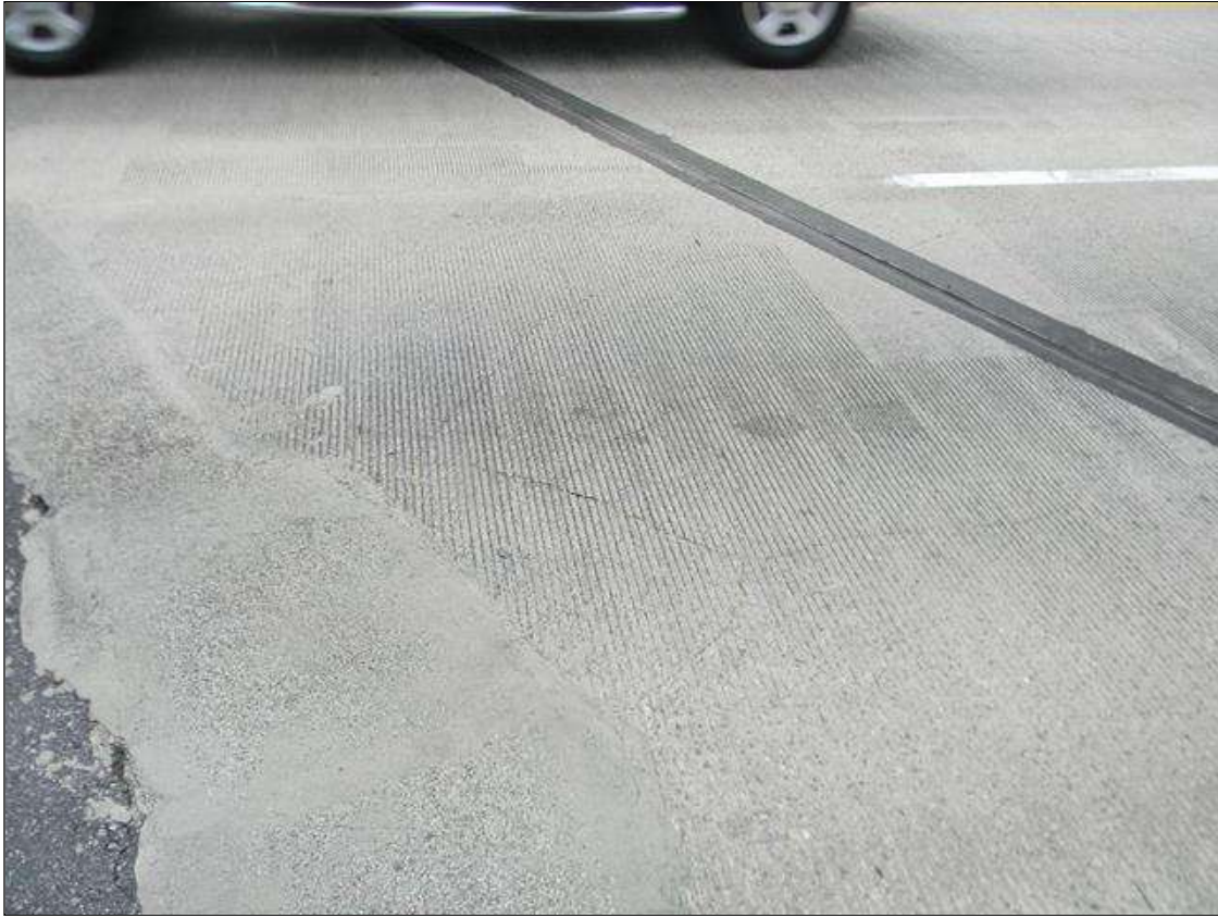
Approach 2: LATEX MODIFIED CONCRETE WEARING SURFACE HAS SCATTERED MAP CRACKS.
