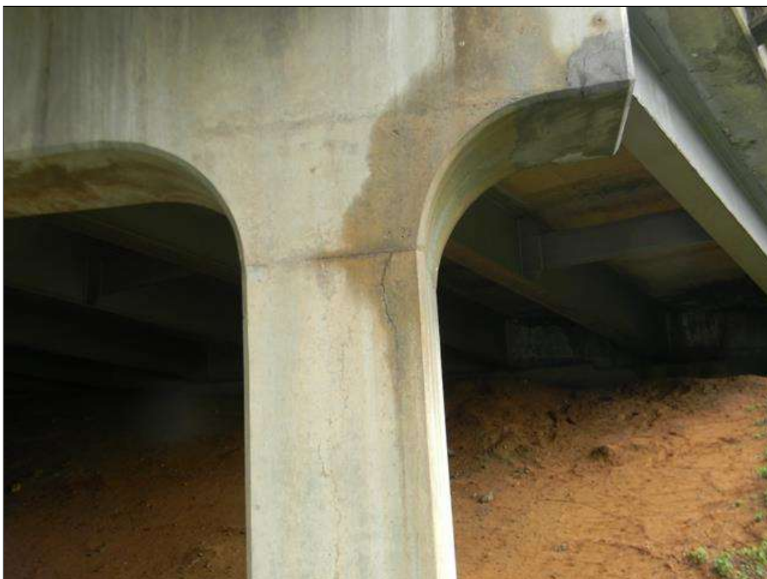
Bent 2 Pile 5: WEST FACE OF THE COLUMN HAS A 3' LONG VERTICAL H/L CRACK JUST BELOW THE HAUNCH.
