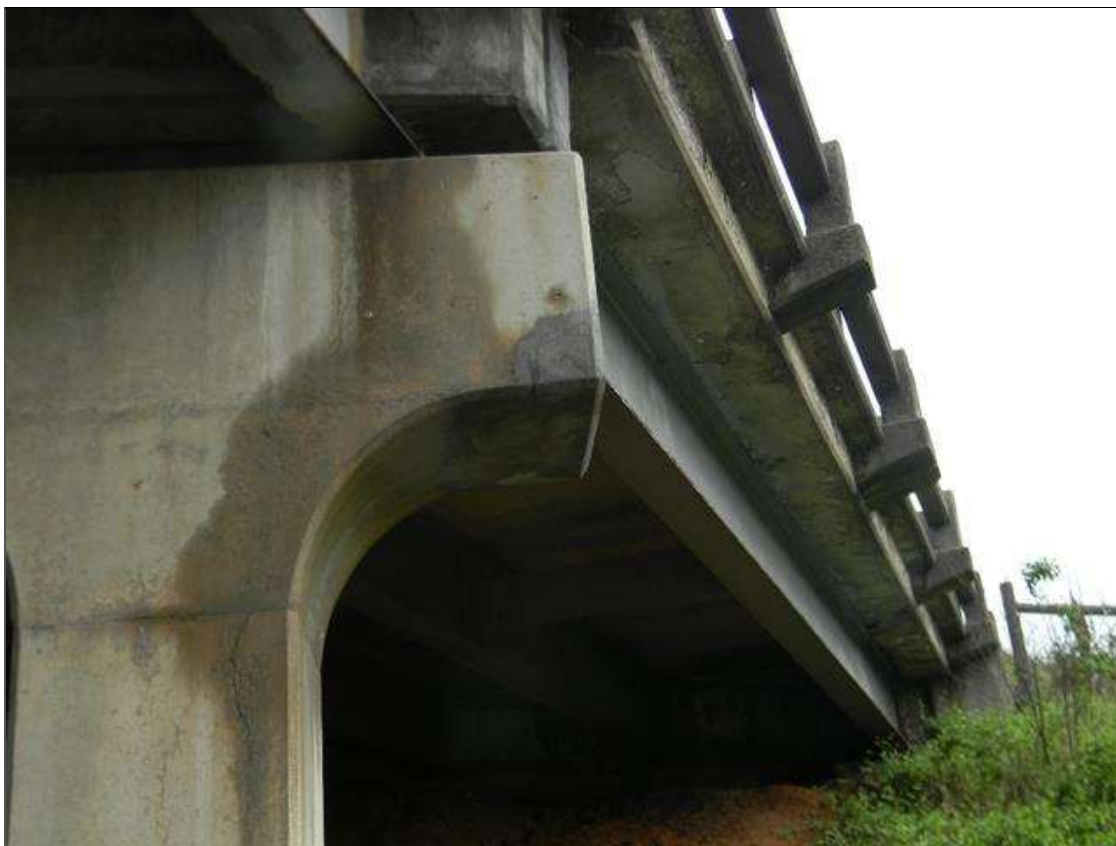
Bent 2 Cap 1: WEST FACE AND RIGHT END OF CAP HAS A PATCH IN GOOD CONDITION. THIS IS CONSIDERED A TEMPORARY REPAIR.
