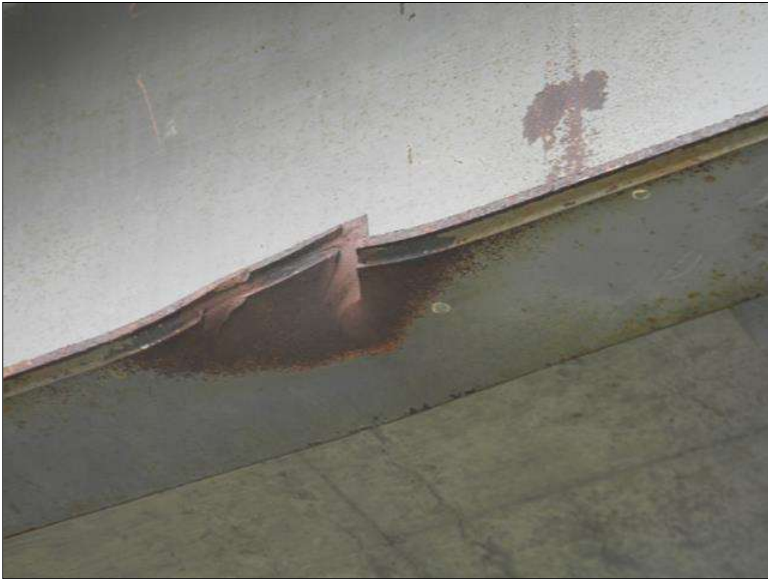
Span 2 Beam 10: IMPACT DAMAGE TO THE RIGHT BOTTOM FLANGE AT 18' 3" FROM THE FACE OF BENT 2 RESULTING IN A TEAR IN THE FLANGE AND COVER PLATE. THERE IS A 9/16" CRACK RUNNING EASTWARD FROM THE TOP OF THE TEAR. THE BOTTOM FLANGE IS BENT 1" TOWARD THE NORTH IN THIS AREA. SEE DAMAGE INSPECTION DATED 8/1/2011 FOR FURTHER DETAILS.
