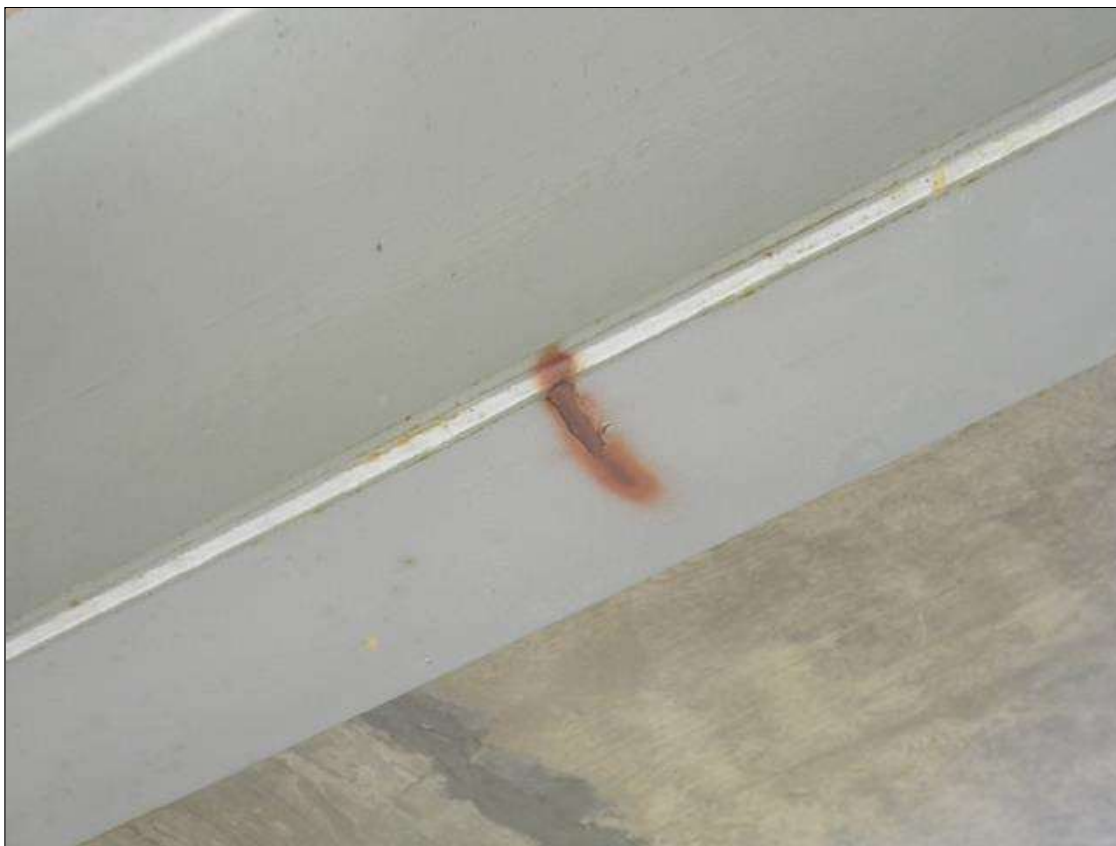
Span 2 Beam 9: RIGHT BOTTOM FLANGE HAS A 4" LONG X 1" WIDE X 1/16" DEEP GOUGE DUE TO IMPACT AT 18" 6" FROM THE FACE OF BENT 2 CAP. SEE DAMAGE INSPECTION DATED 8/1/2011 FOR FURTHER DETAILS.
