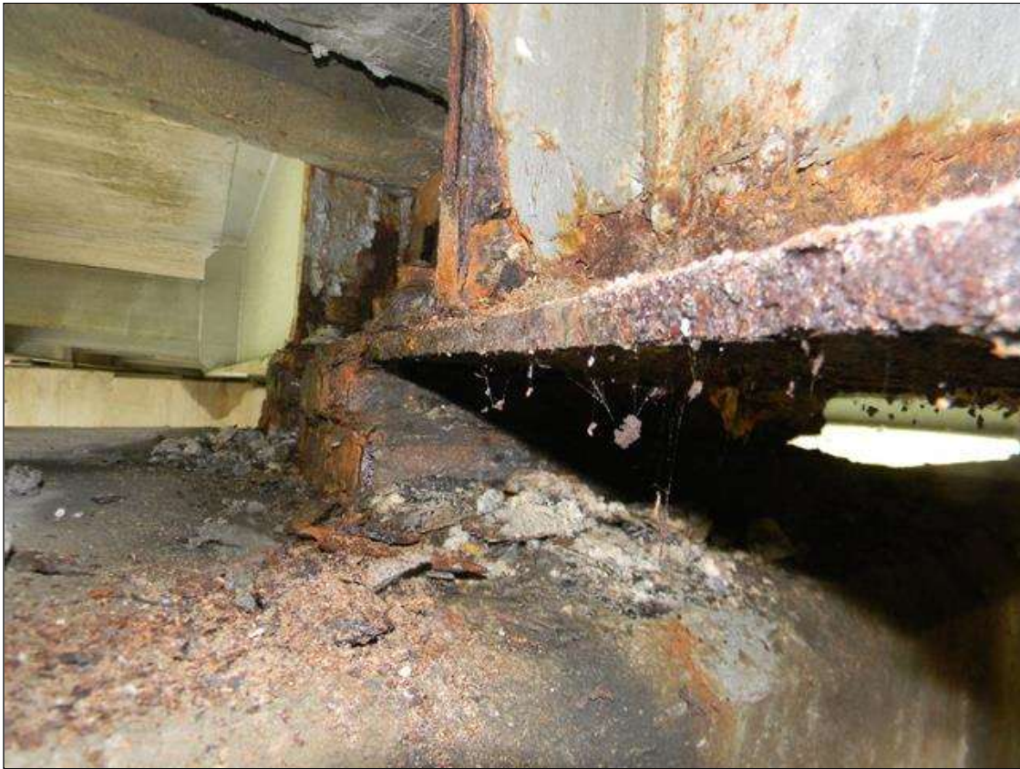
Span 1 Beam 3: LEFT BOTTOM FLANGE AT BENT 1 IS DOWN TO 7/16" FROM THE ORIGINAL 9/16" THICKNESS FOR 1' 3" LONG STARTING AT THE END X FULL WIDTH. A PRIORITY MAINTENANCE IS BEING ISSUED FOR THIS BEAM.
