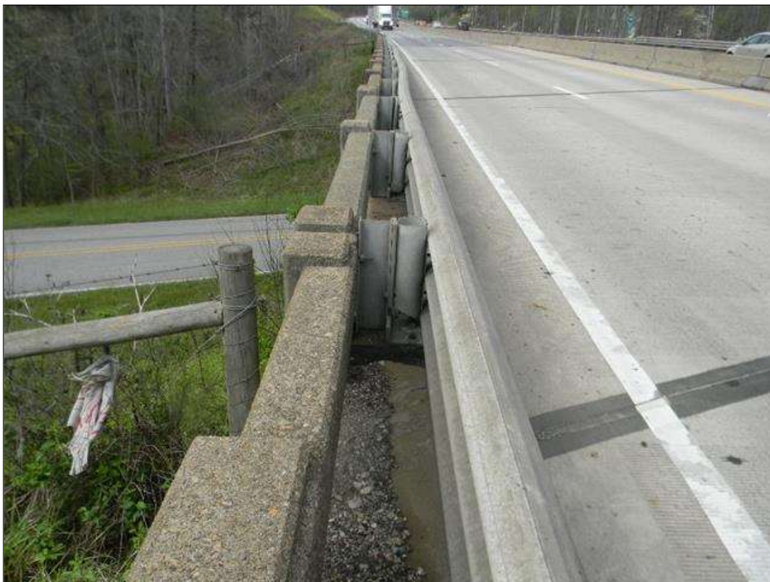
TRI-BEAM RETROFIT RAIL WAS INSTALLED INSIDE OF THE ORIGINAL RAILS IN THE PAST.
