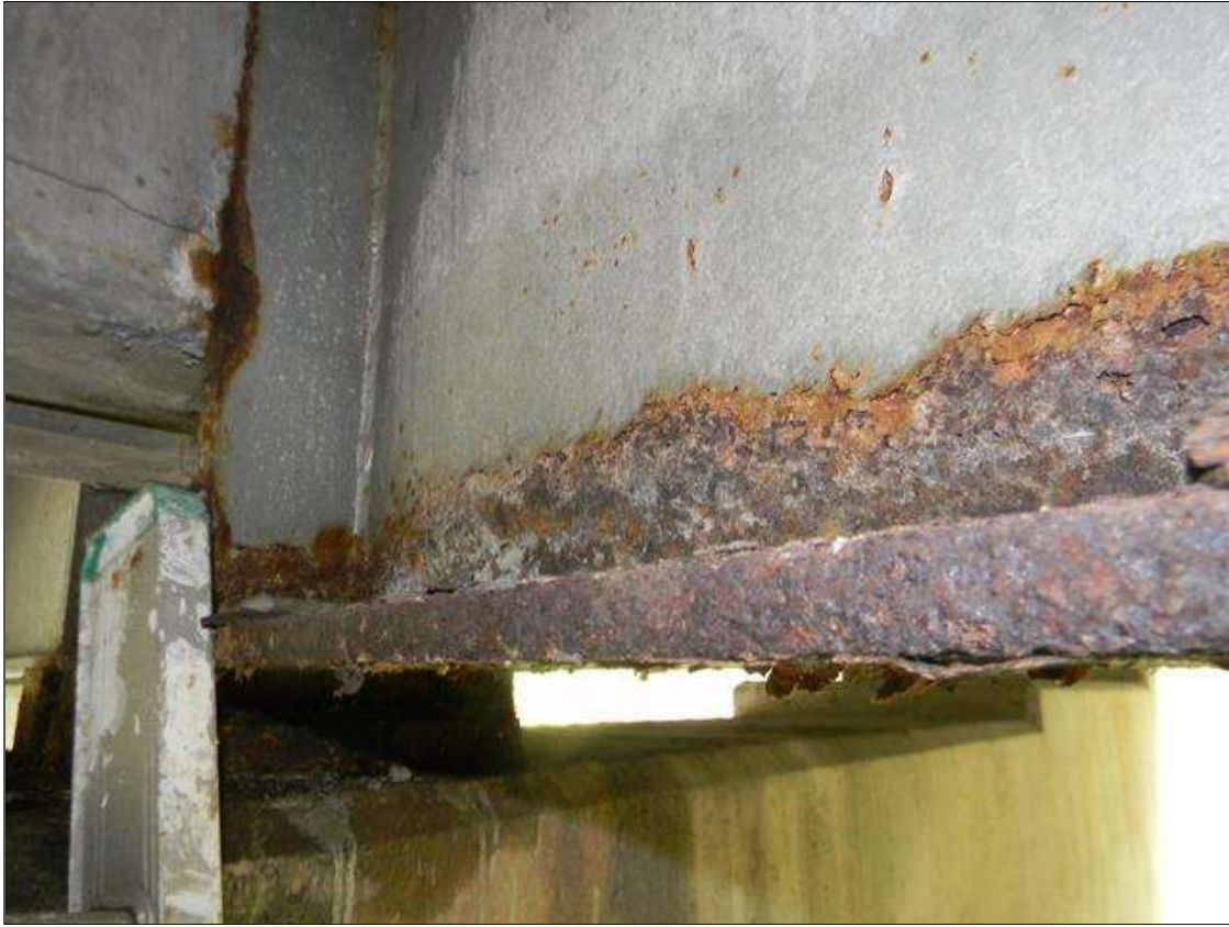
Span 3 Beam 3: RIGHT BOTTOM FLANGE AT BENT 2 HAS FLAKING SURFACE CORROSION WITH NO SIGNIFICANT LOSS FOR 6' LONG.
