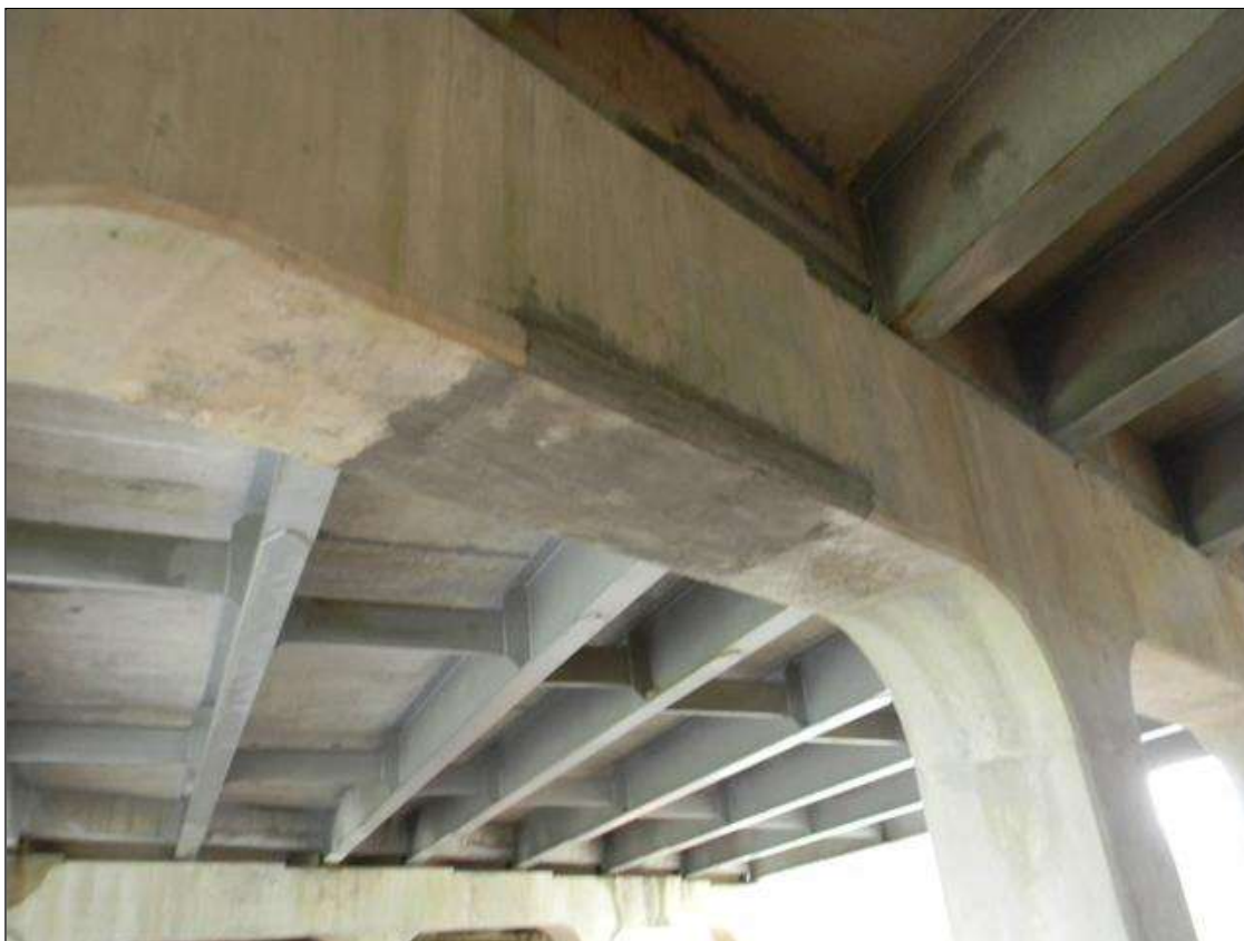
Bent 1 Cap 1: CAP HAS SEVERAL PATCHES IN GOOD CONDITION. THESE ARE CONSIDERED TEMPORARY REPAIRS.
