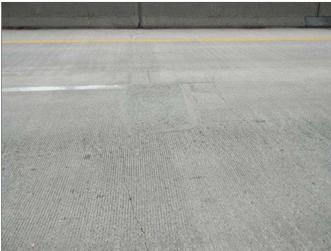
Span 3 Wearing Surface: 2' LONG X 4' WIDE PATCH IN THE WEARING SURFACE IN THE WESTBOUND RIGHT LANE. PATCH IS IN GOOD CONDITION.
