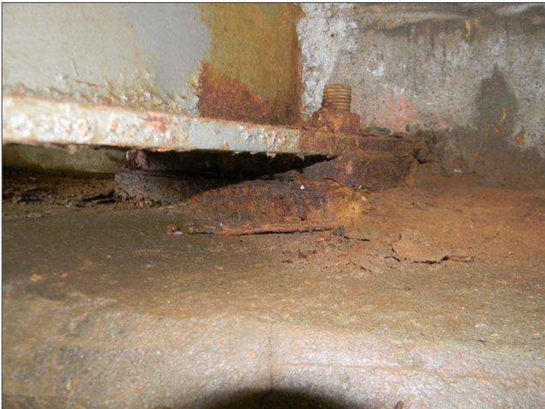
Span 3 Beam 10 Far Bearing: LOSS OF PAINT ALLOWING SURFACE CORROSION OVER THE ENTIRE BEARING.
