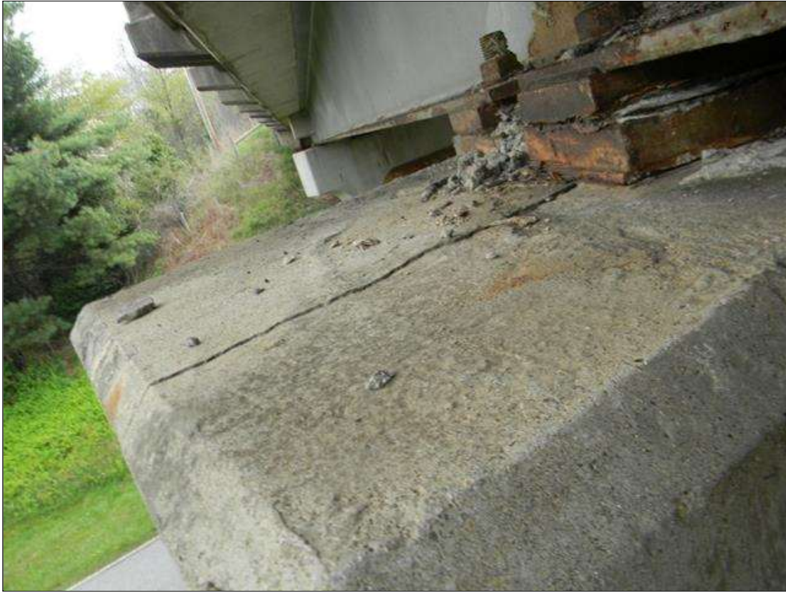
Bent 1 Cap 1: LEFT END OF BENT 1 CAP HAS A CRACK WITH A 30" WIDE X 14" HIGH X 12" DEEP SPALL FORMING UNDER BEAM 1 BEARING. THE CRACK RUNS UNDER THE CENTER OF THE BEARING MASONRY PLATE. A PRIORITY MAINTENANCE WAS ISSUED LAST INSPECTION AND IS BEING RE-ISSUED FOR THIS SPALL.
