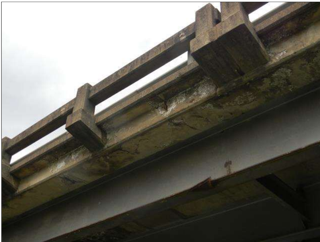
Span 2 Deck: SCATTERED SPALLS, SOME WITH EXPOSED REBAR, ALONG THE UNDERSIDE OF THE OVERHANGS.
