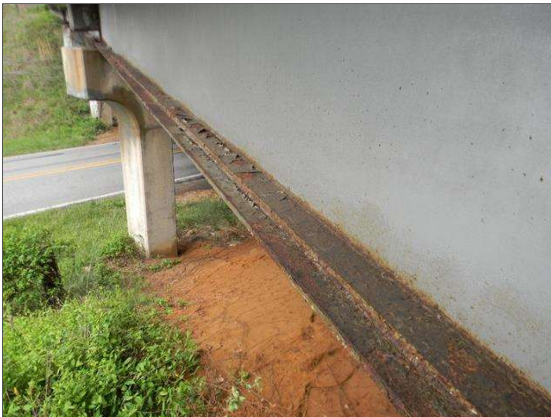
Span 2 Beam 10: PEELING PAINT ALONG THE TOP OF THE BOTTOM FLANGE ALLOWING SURFACE CORROSION.
