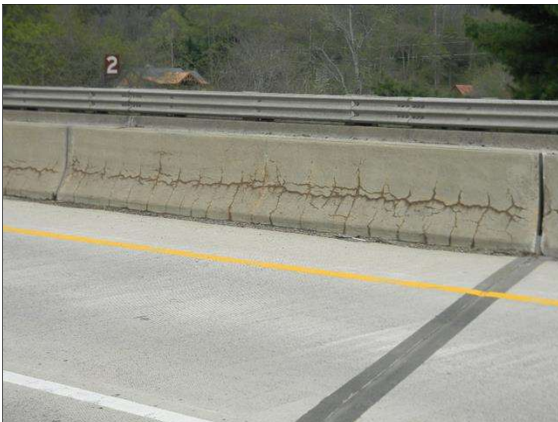
Span 2 Median Rail: H/L MAP AND LONGITUDINAL CRACKS ESPECIALLY ON THE SOUTH FACE.
