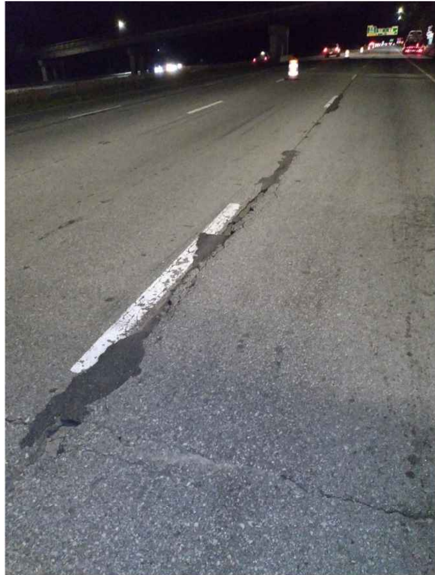
#11: REFLECTIVE CRACKING AT LONGITUDINAL JOINT, SEVERE JOINT DEGRADATION, PATCHED, TYPICAL
