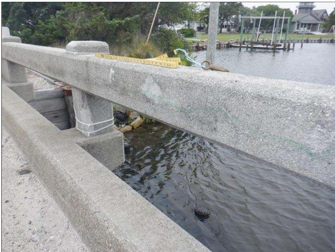
Span 1 Left Bridge Rail: CRACKED TO .062 INCH AND DELAMINATED ALONG INSIDE OF TOP RAIL X FULL LENGTH OF SPAN.
