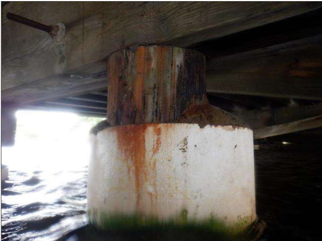
ALL PILES ARE JACKETED WITH CONCRETE FROM 1 FOOT ABOVE MUDLINE TO 8-10 INCHES BELOW CAP. CONCRETE JACKET REPAIRS ARE IN POOR CONDITION WITH LIMITED COVERAGE.
