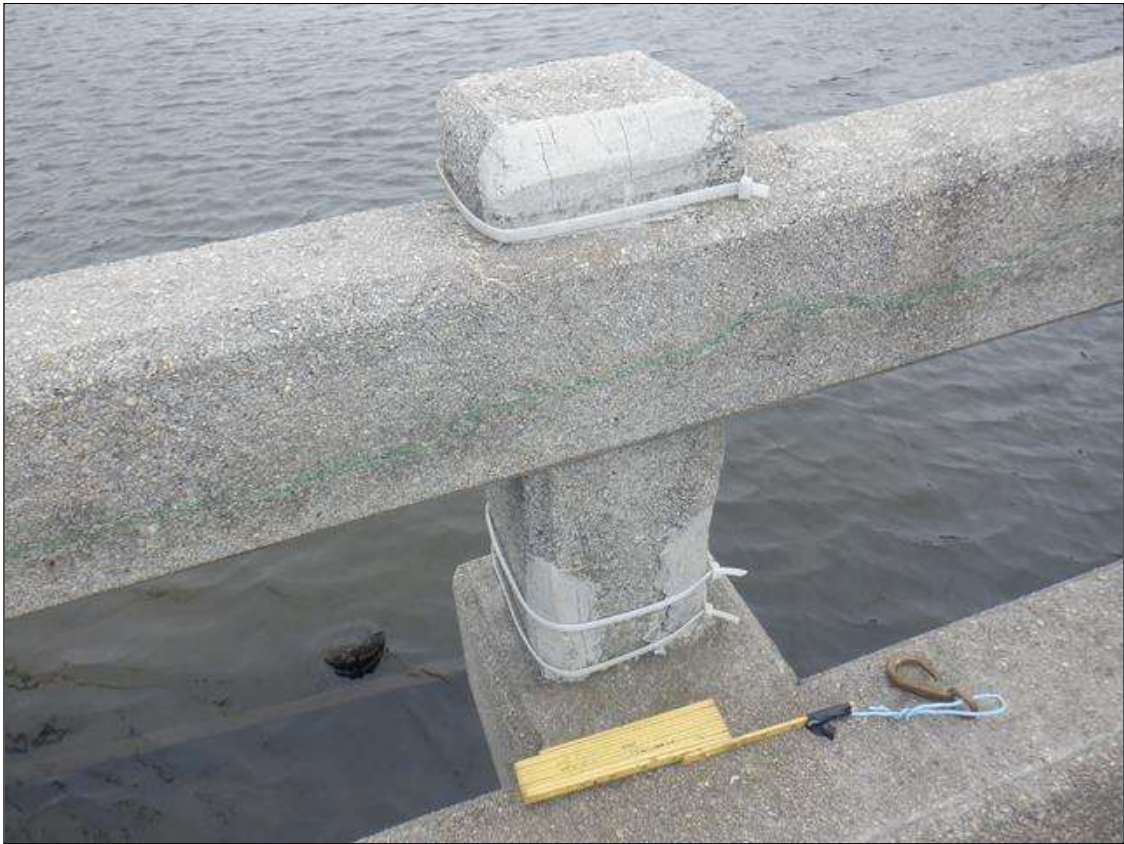
Span 1 Left Bridge Rail: PATCHED AREAS ON RAIL POST 1 2 AND 3.
