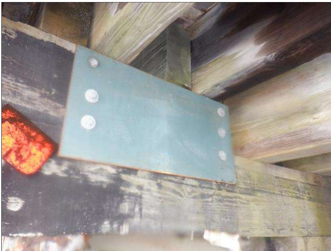
Bent 2 Cap: PEDESTRAIN WALKWAY SUBCAP HAS BEEN REPAIRED WITH A STEEL SPLICE PLATE.
