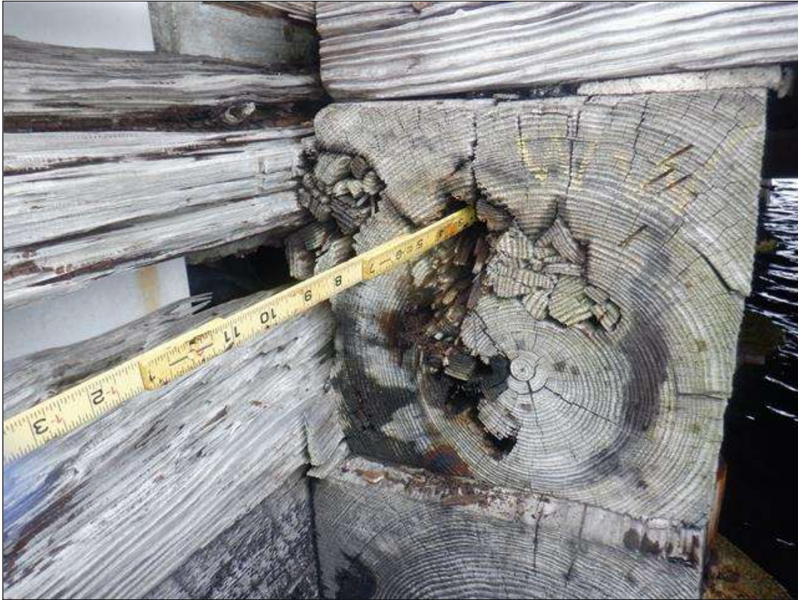
End Bent 1 Cap: PAR- PEDESTRAIN WALKWAY SUBCAP HAS DECAY ON THE EAST END CENTER OF CAP. 8 INCH DIAMETER X 4 INCHES DEEP
