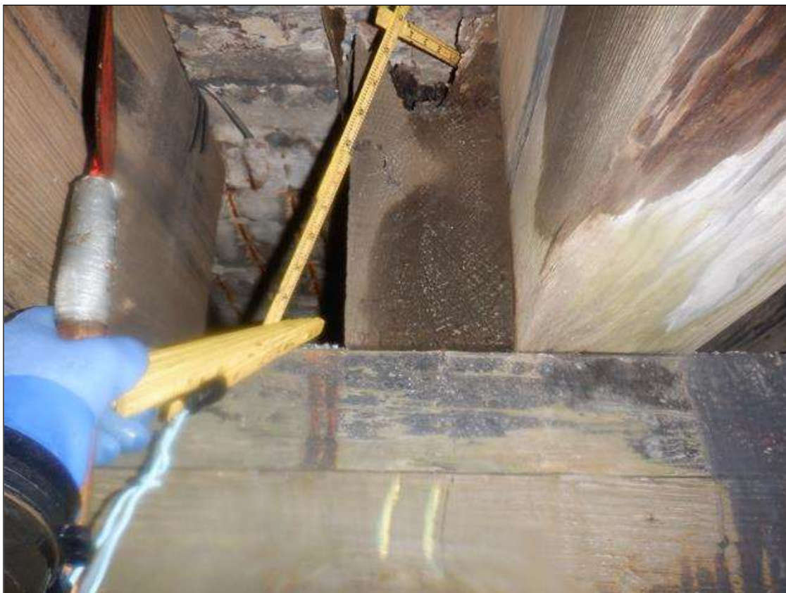
Span 1 Beam 11: PAR- DECAYED ON END OVER BENT 1, 5 INCHES TALL X 6 INCHES WIDE X 6 INCHES DEEP.
