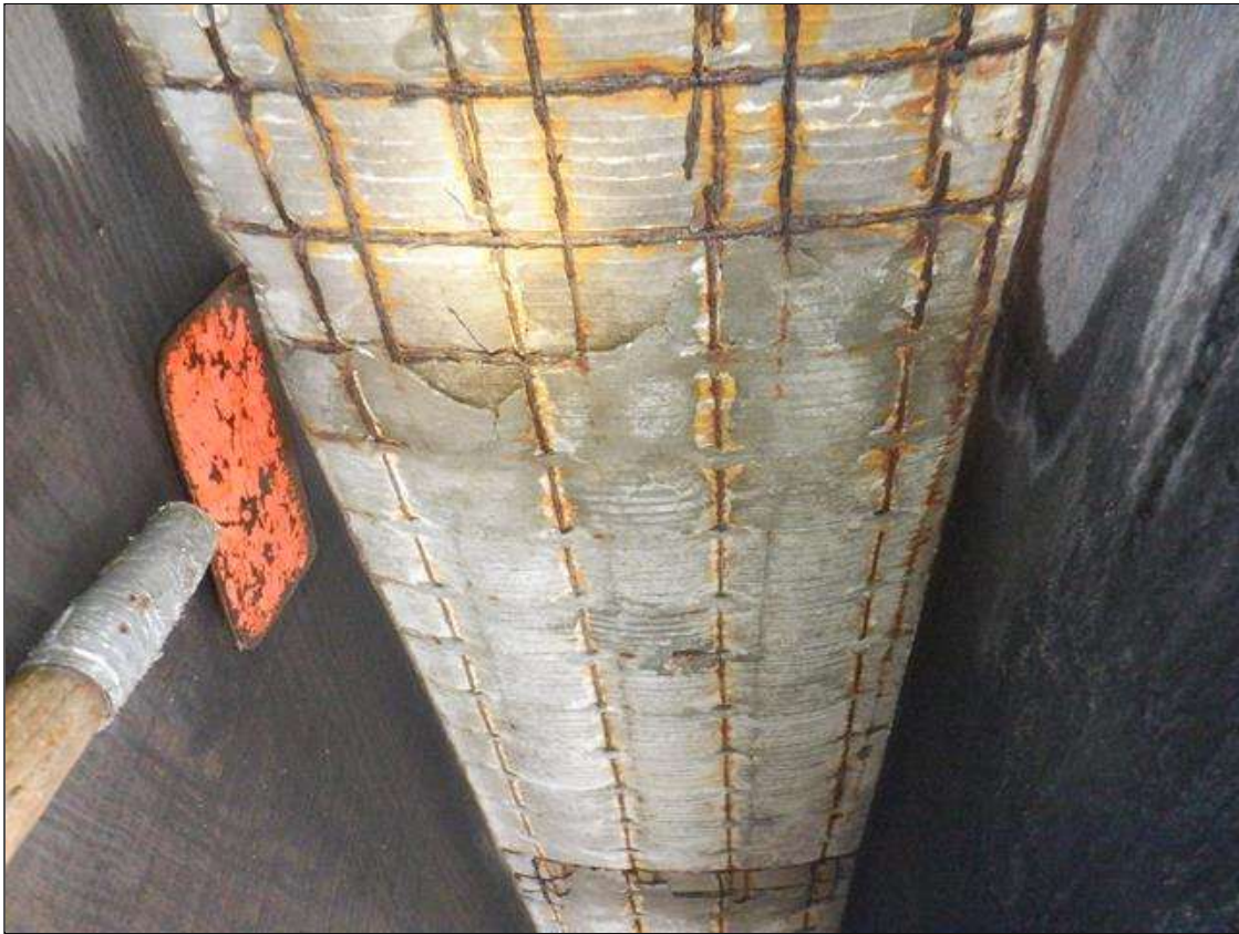
BOTTOM OF DECK COVERED IN WIRE AND PAPER
