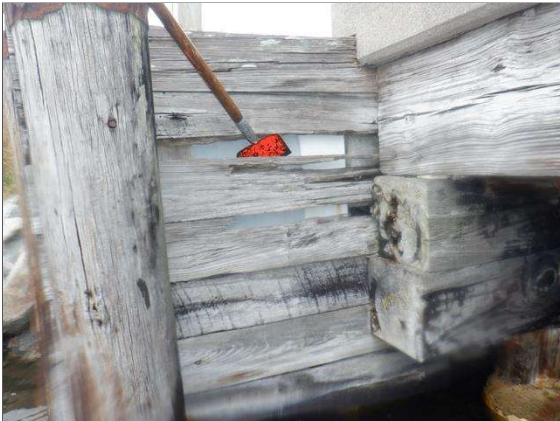
VINYL SHEETING HAS BEEN DRIVEN BEHIND SOUTH EAST TIMBER ABUTMENT. GOOD CONDITION
