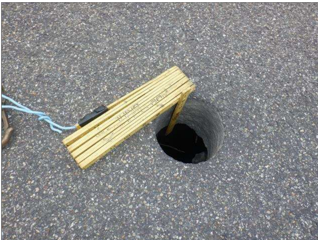
Span 3 Deck: PAR- 4 INCH DIAMETER HOLE THROUGH DECK IN SOUTH BOUND LANE.
