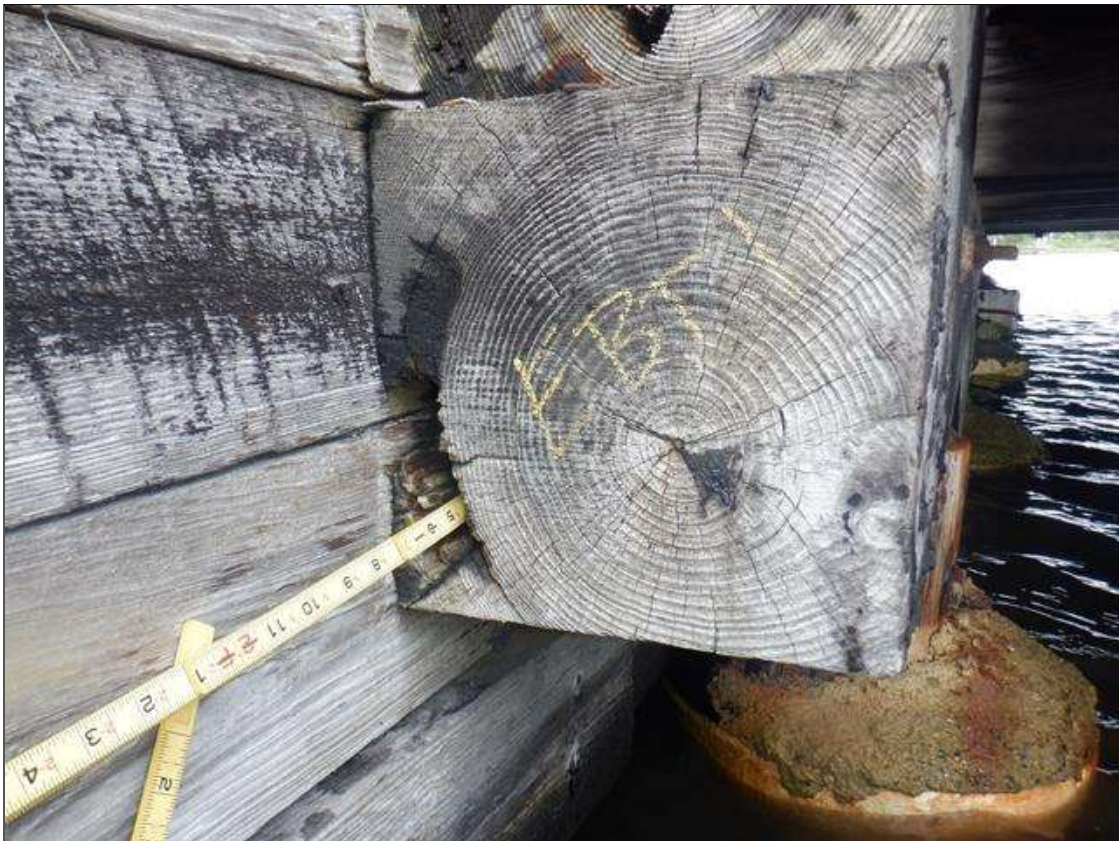
End Bent 1 Cap 1: PAR: EAST END DECAYED FROM END BACK 16 INCHES, 5 INCHES TALL X 2 INCHES WIDE .
