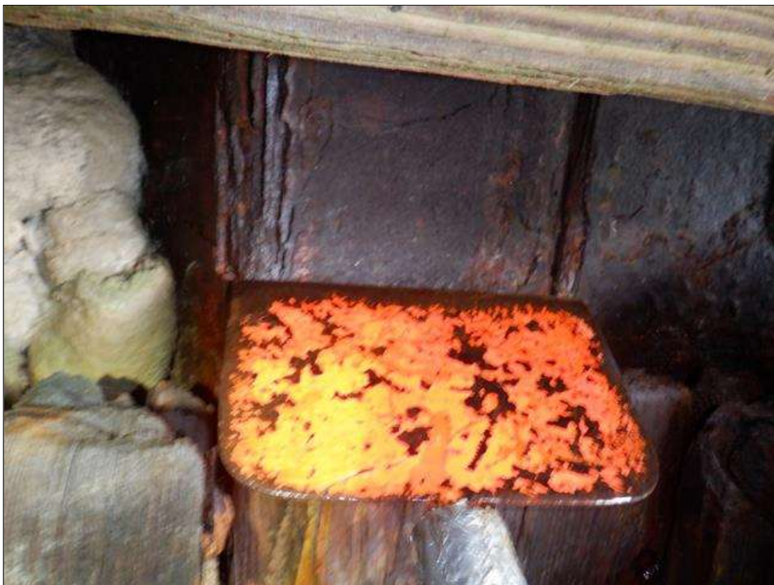
RUST AND SCALE ON SHEET PILE OLD TIMBER ABUTMENT. BOTH END BENT 1 AND 2.
