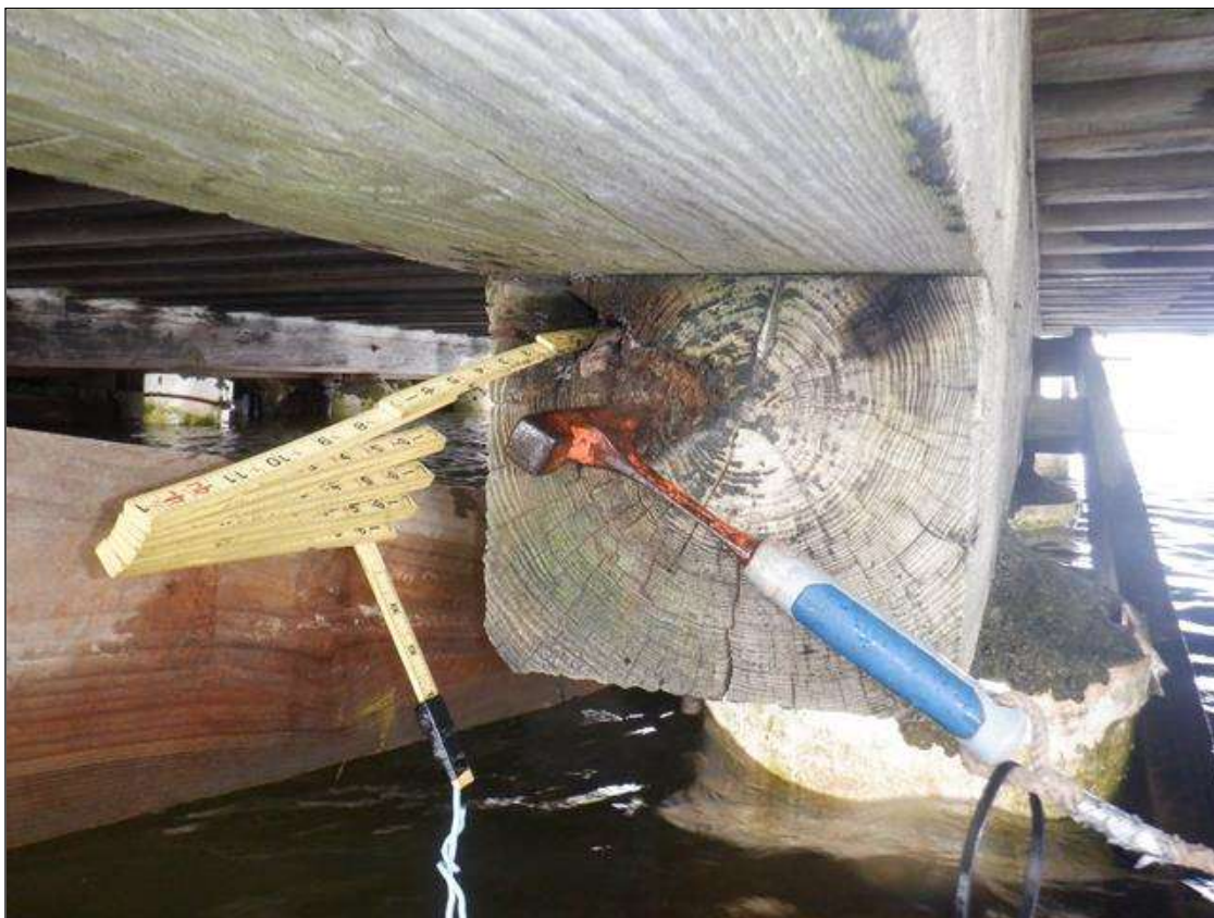
Bent 1 Cap: SUBCAP HAS DECAY ON EAST END TOP CORNER, 4 INCH DIAMETER X 14 INCHES DEEP
