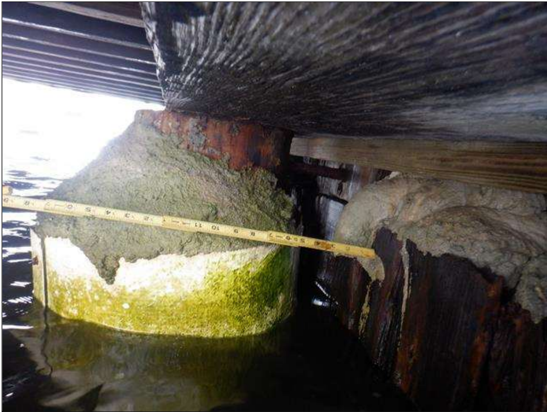
CONCRETE JACKET REPAIRS ARE IN POOR CONDITION WITH LIMITED COVERAGE. ALL PILES HAVE CHECKS TO .125 INCH WIDE, SOFT TO .50 INCH DEEP WHERE TIMBER PILE IS EXPOSED.
