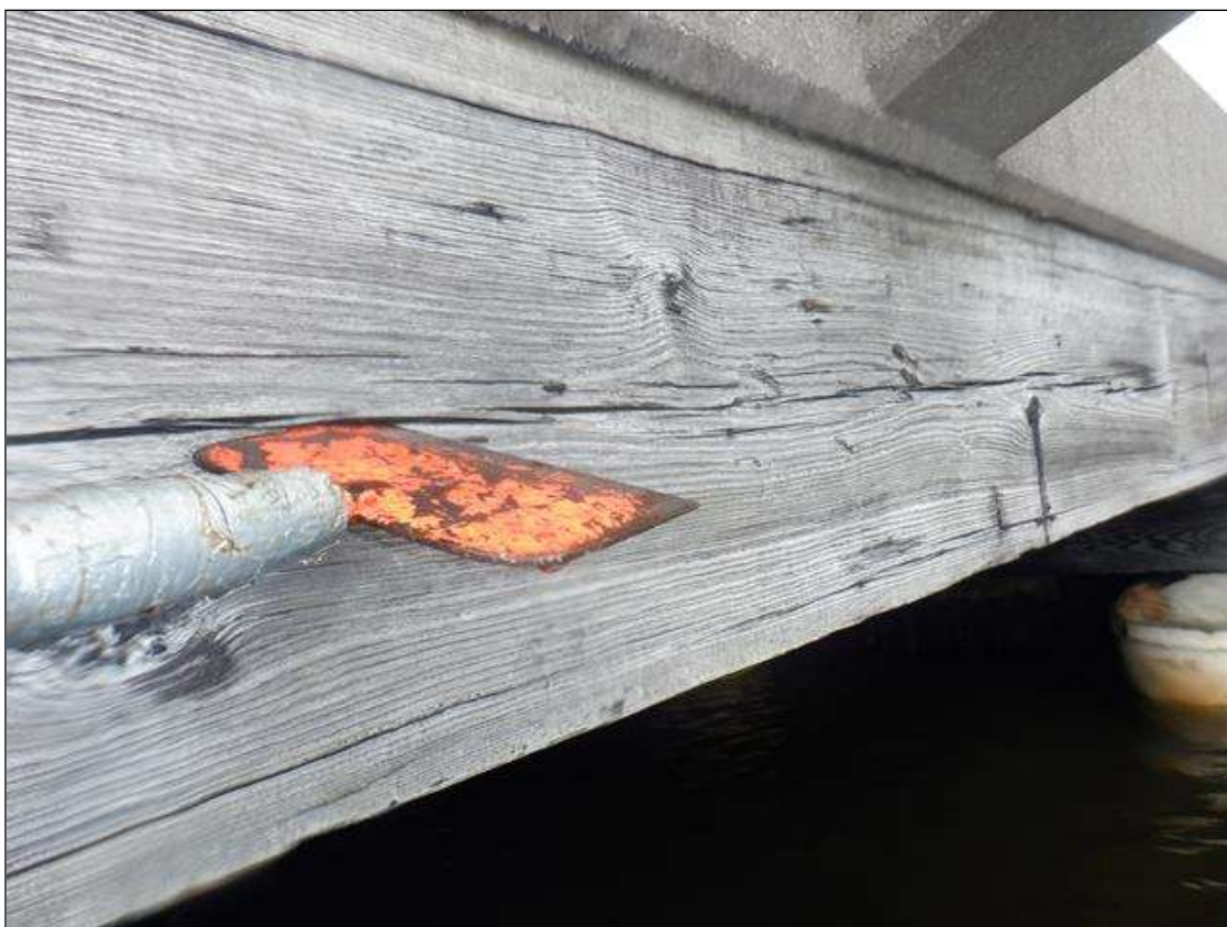
EXTERIOR JOISTS HAVE CHECKS TO .25 INCH WIDE, WEATHERED, AND SOFT TO .50 INCH DEEP
