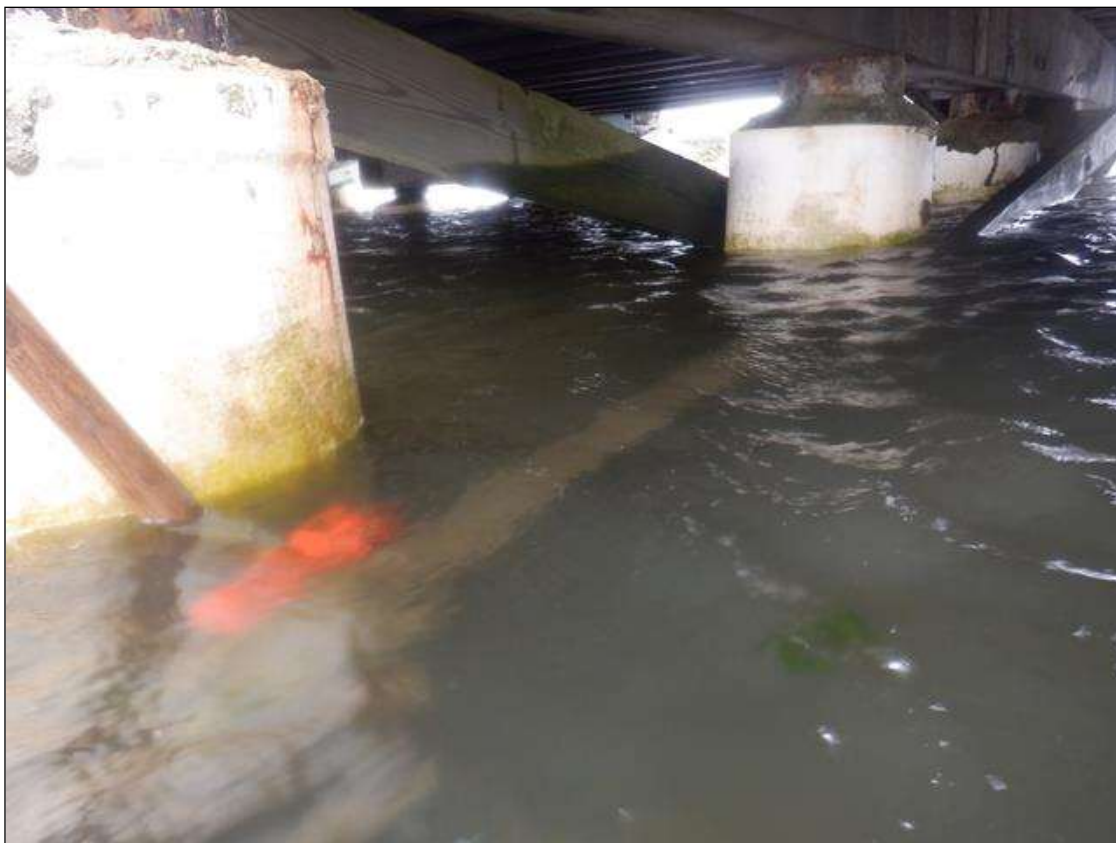
Bent 1 Pile 1: PAR: X-BRACING DECAYED AND DETACHED FROM PILE.
