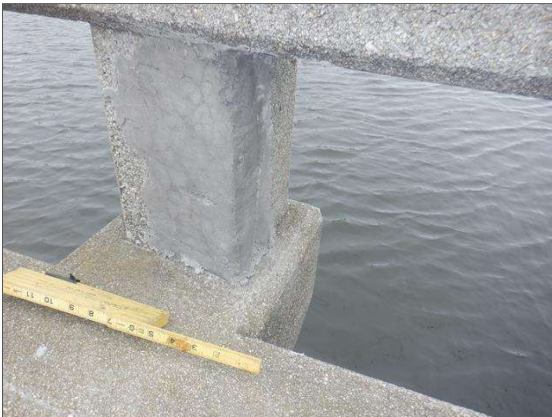
Span 3 Left Bridge Rail: PAR: RAIL POST 2 HAS A FAILED PATCH WITH EXPOSED REINFORCING STEEL 2 INCH DIAMETER. AREA HAS BEEN REPAIRED.
