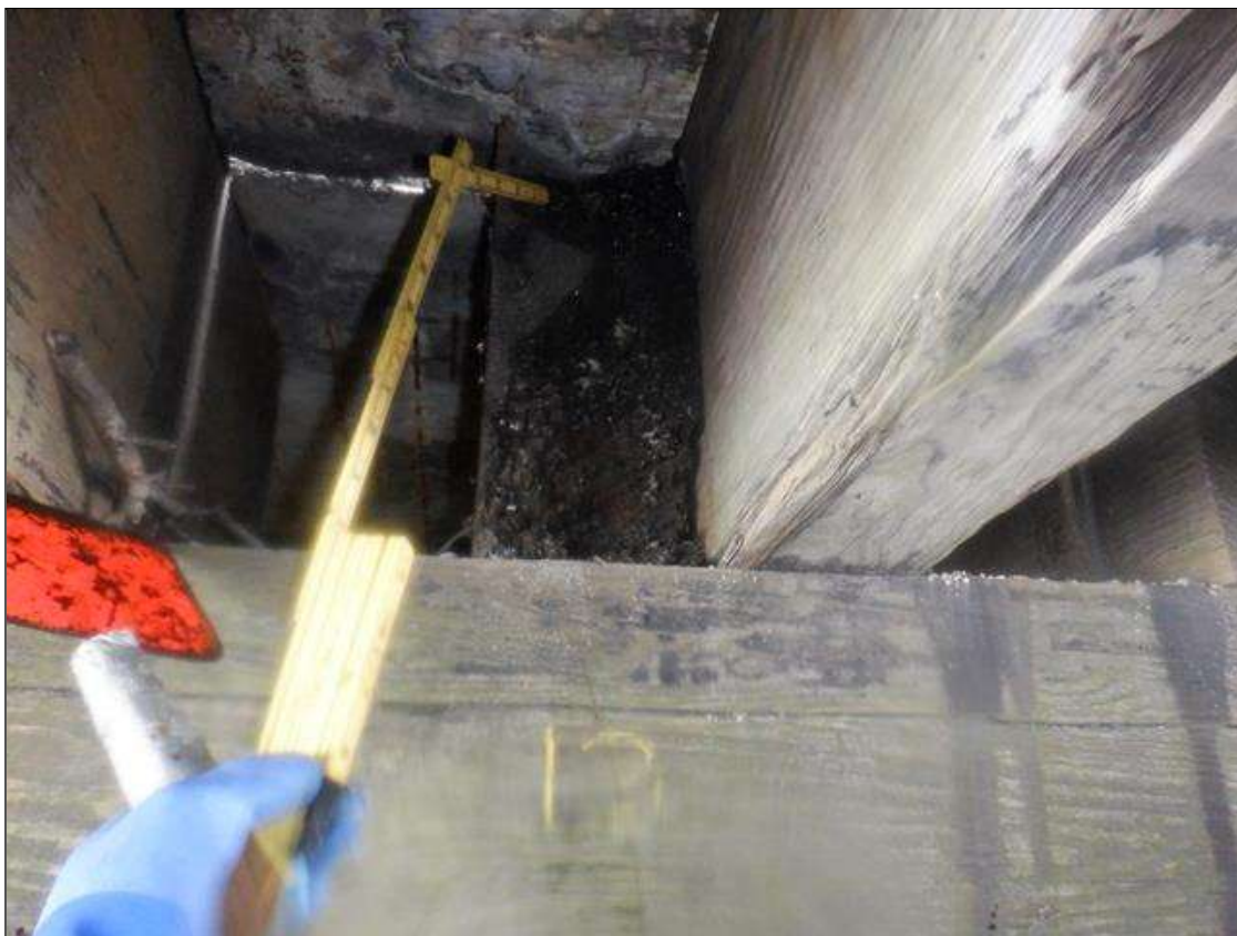
Span 1 Beam 13: PAR- DECAYED ON END OVER BENT 1, 4 INCHES TALL X 6 INCHES WIDE X 5 INCHES DEEP.
