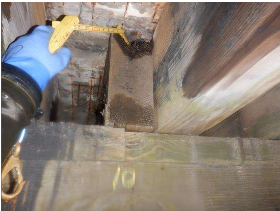
Span 1 Beam 10: PAR- DECAYED ON END OVER BENT 1, 4 INCHES TALL X 6 INCHES WIDE X 5 INCHES DEEP.
