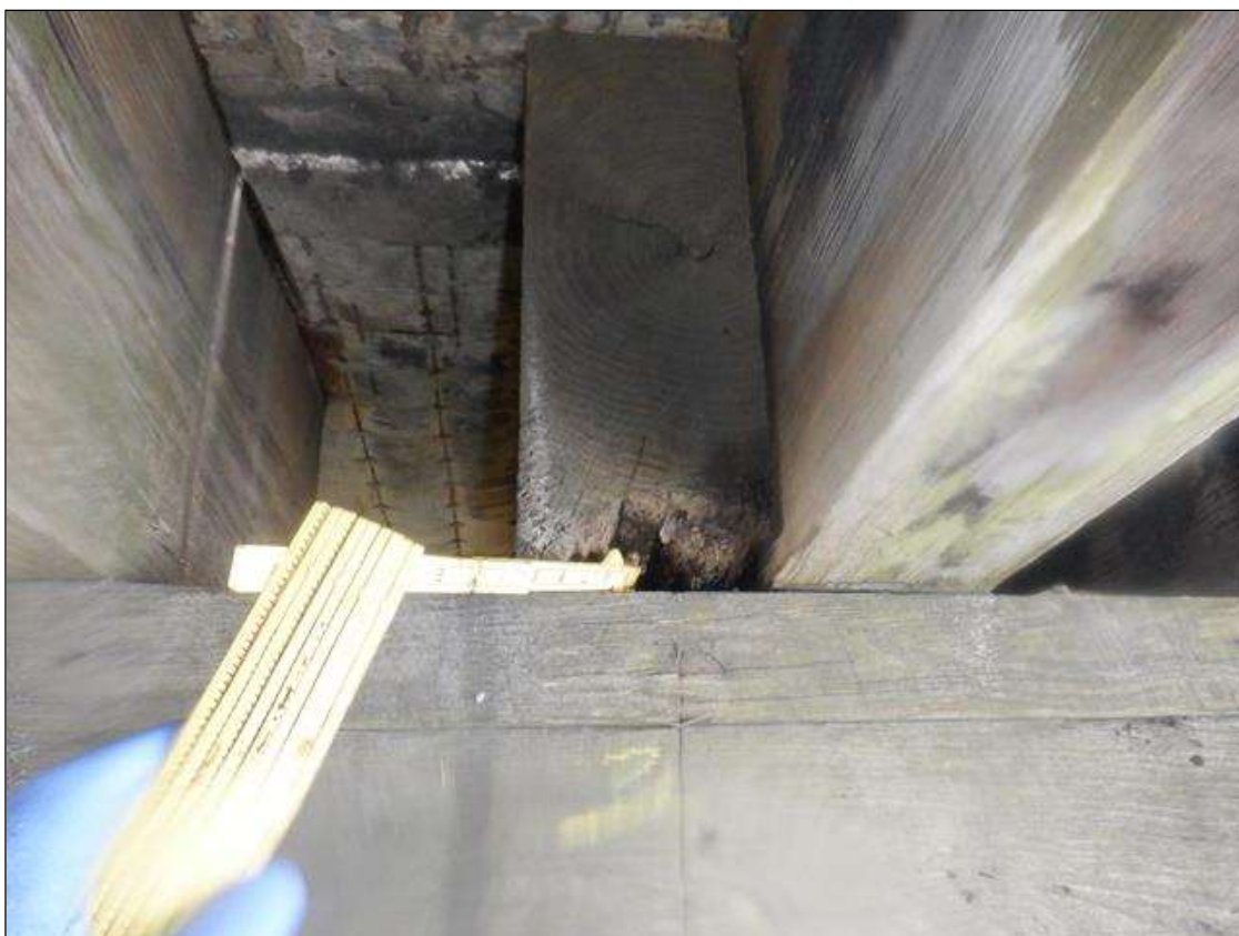
Span 1 Beam 3: PAR- DECAYED ON END OVER BENT 1, 4 INCHES TALL X 6 INCHES WIDE X 5 INCHES DEEP.
