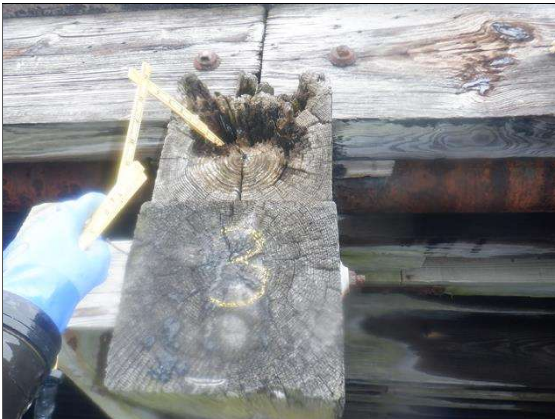
Bent 3 Cap: PAR: PEDESTRAIN WALKWAY SUBCAP HAS DECAY ON EAST END IN CENTER. 9 INCH DIAMETER X 9 INCHES DEEP.
