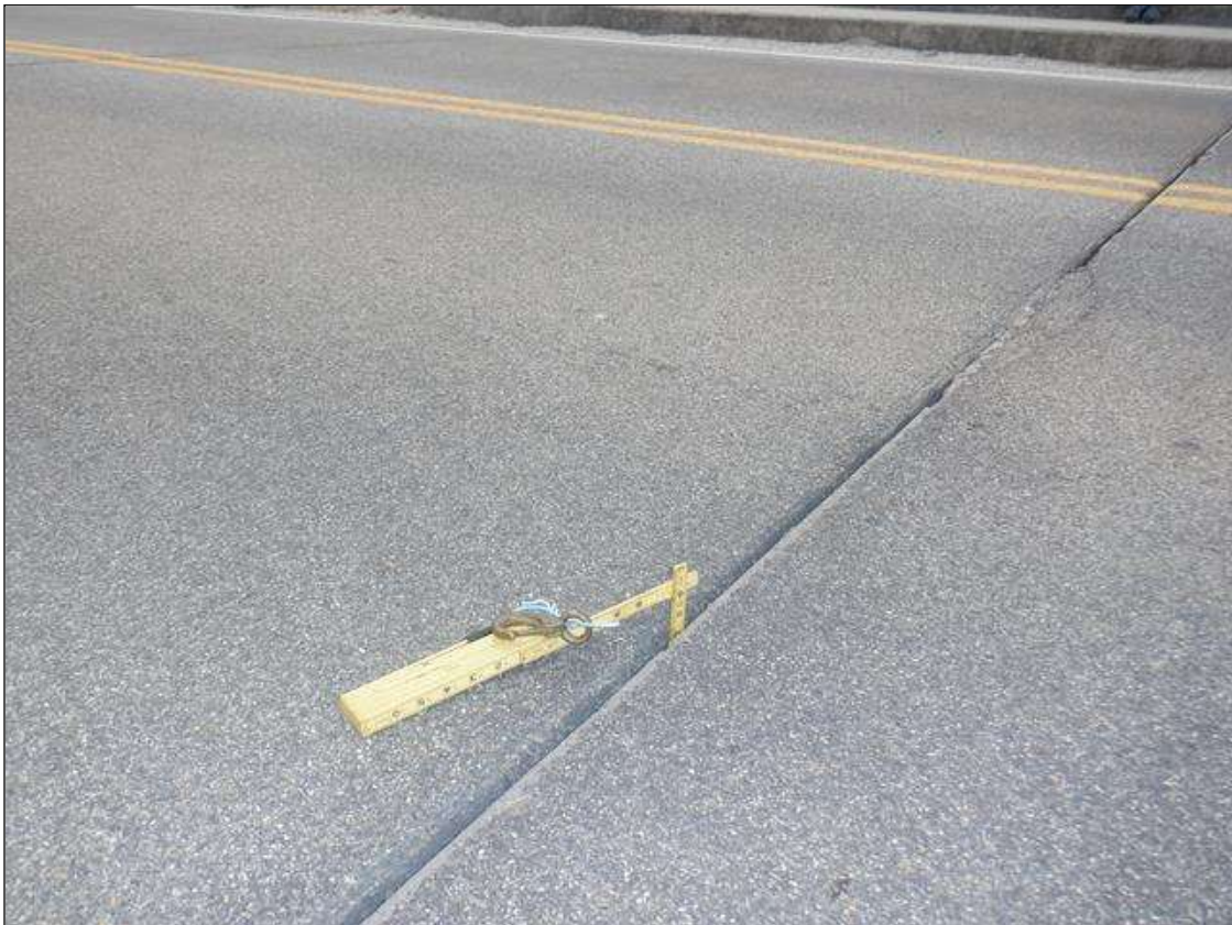
Span 2 Expansion Joint: JOINT HAS A 1 INCH GAP WHERE JOINT MATERIAL IS MISSING, ALLOWING WATER TO DRAIN ON SUPERSTRUCTURE AND SUBSTRUCTURE COMPONENTS.
