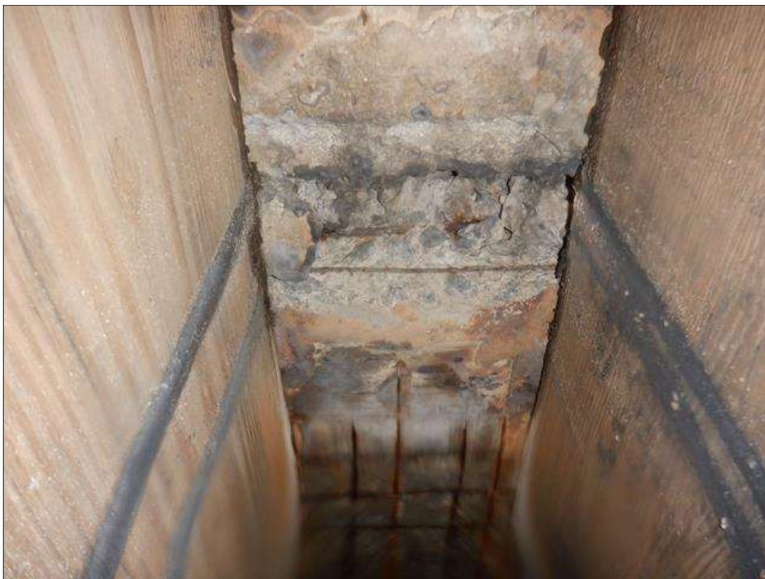
OPEN AREA ON EXPANSION JOINT ALLOWING DEBRIS AND WATER LEAKAGE THROUGH.
