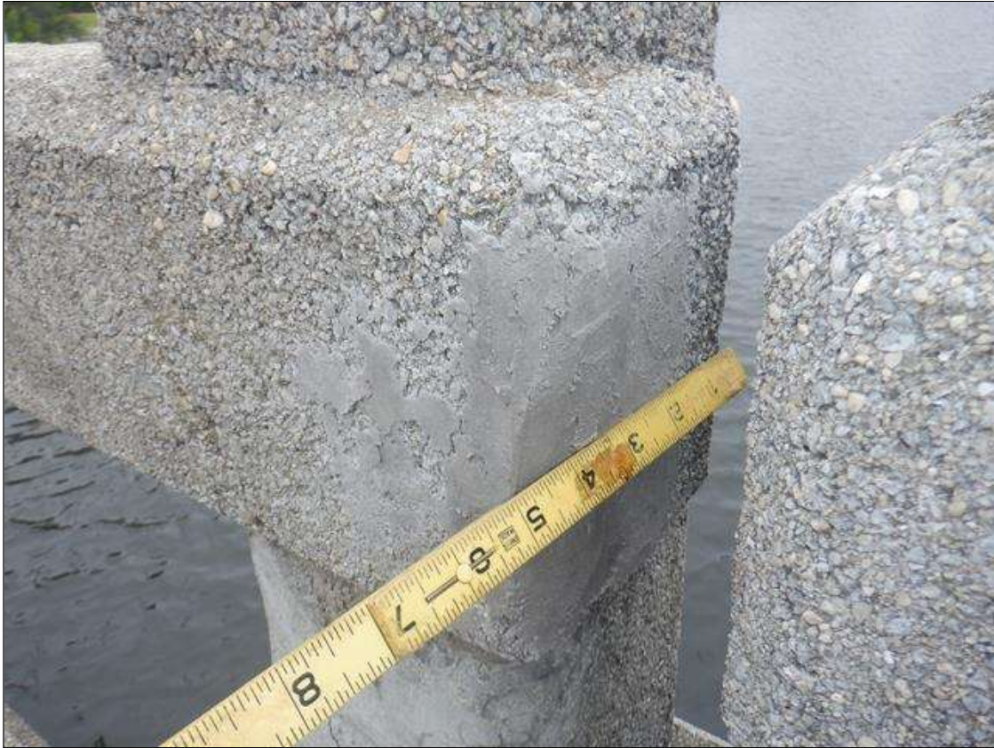
Span 2 Left Bridge Rail: PAR: RAIL OVER POST 3 HAS A 2 INCH X 3 INCH CORNER SPALL EXPOSING REINFORCING STEEL. AREA HAS BEEN REPAIRED
