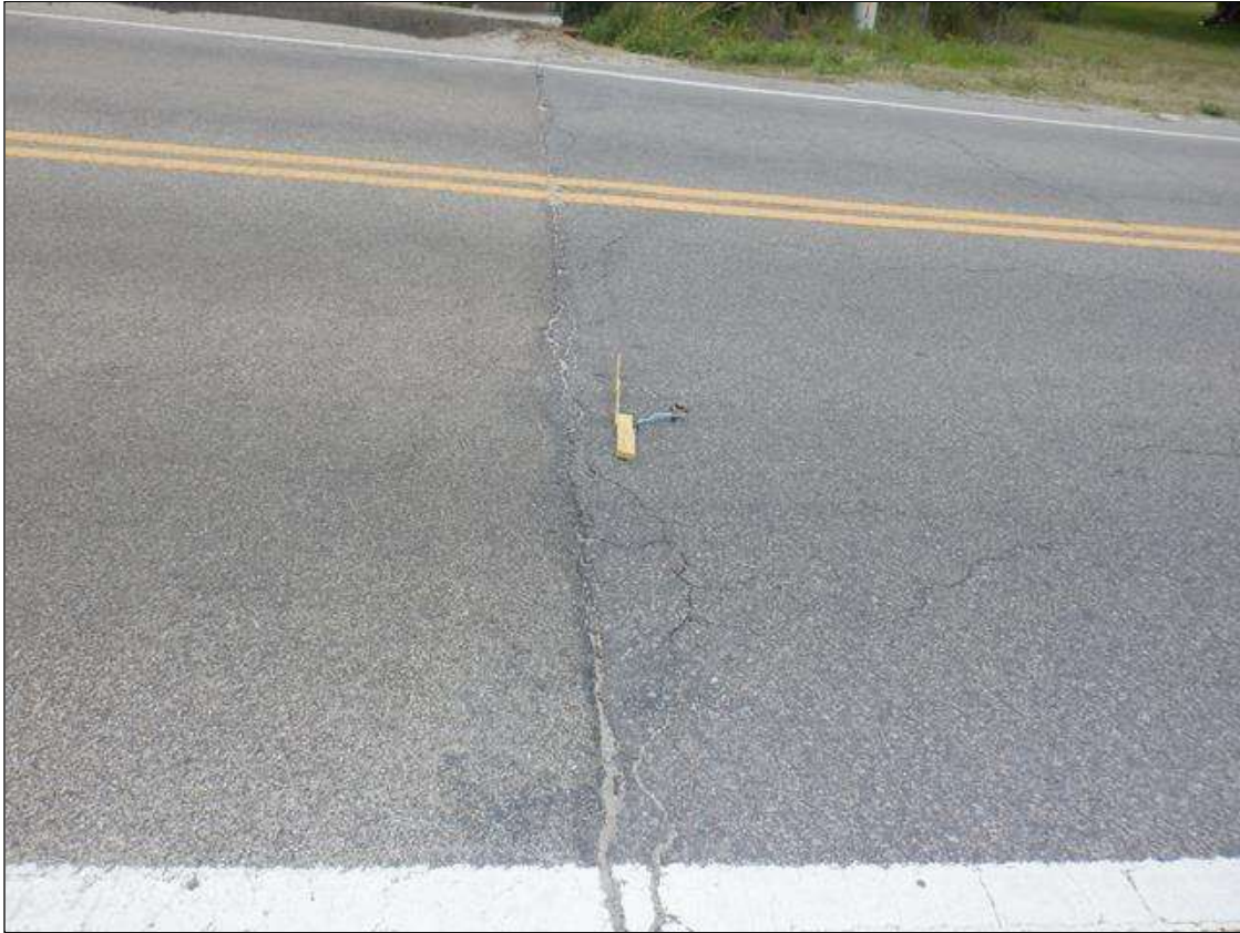
Span 5 Wearing Surface: CRACKED TO .50 INCH, SPALLED TO 1 INCH X FULL WIDTH OF ROADWAY OVER END BENT 2.
