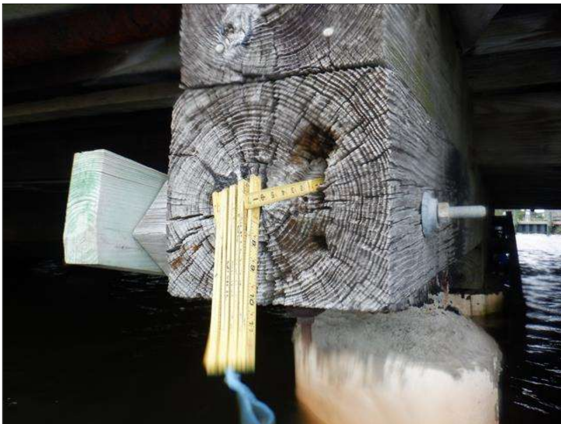
Bent 4 Cap: PAR: EAST END OF CAP AT CENTER, DECAYED AREA 8 INCH DIAMETER X 13 INCHES DEEP.
