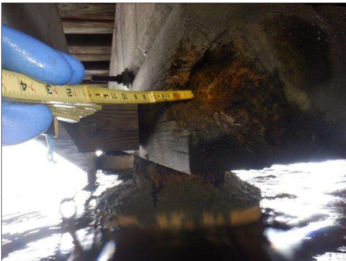
Bent 4 Cap: PAR: BENT 4 SUBCAP WEST END HAS AN AREA OF DECAY 6 INCH DIAMETER X 6 INCHES DEEP.
