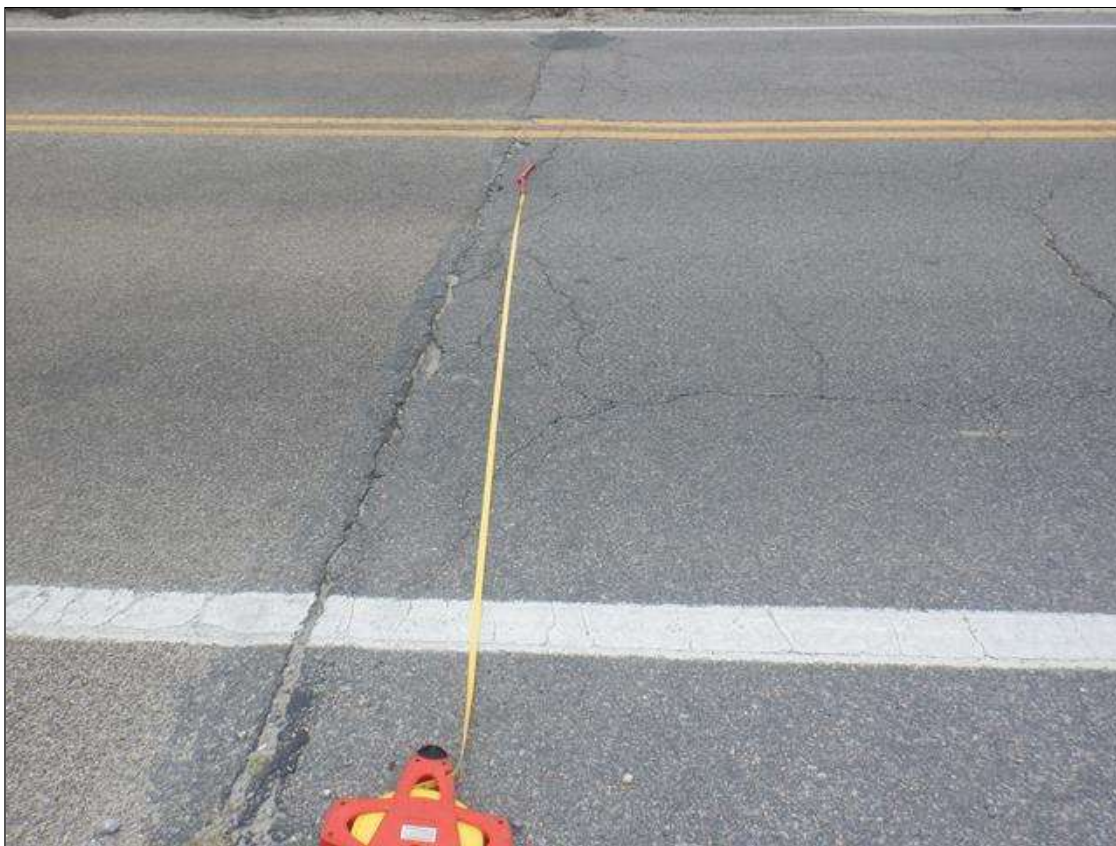
Span 1 Wearing Surface: CRACKED TO .50 INCH, SPALLED TO 3 INCHES WIDE X FULL WIDTH OF ROADWAY OVER END BENT 1.
