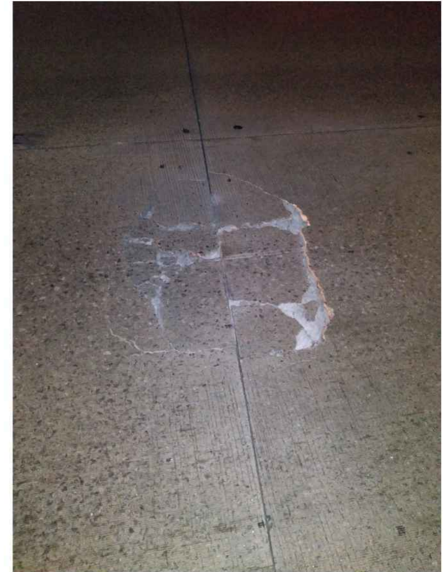
#10: SPALLING CONCRETE/POTHOLE AT LONGITUDINAL JOINT, TYPICAL
