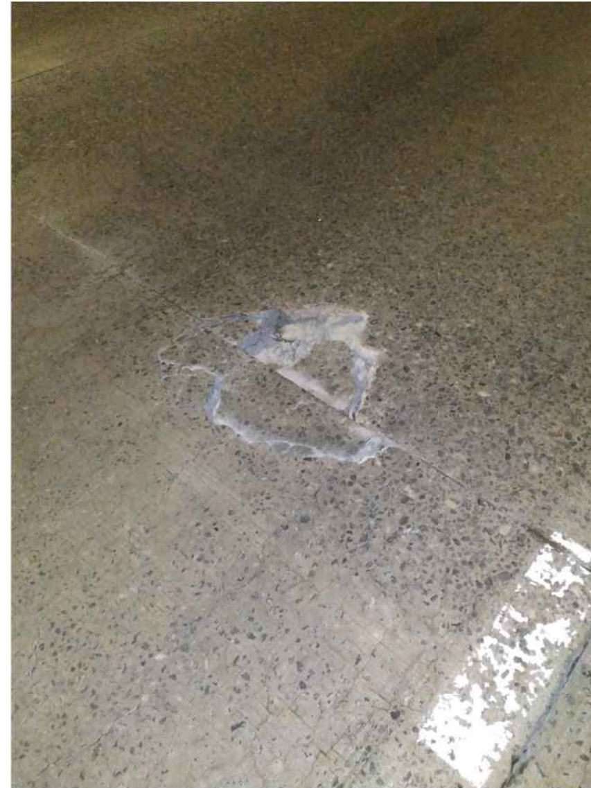
#9: SPALLING CONCRETE/POTHOLE AT TRANSVERSE JOINT, TYPICAL
