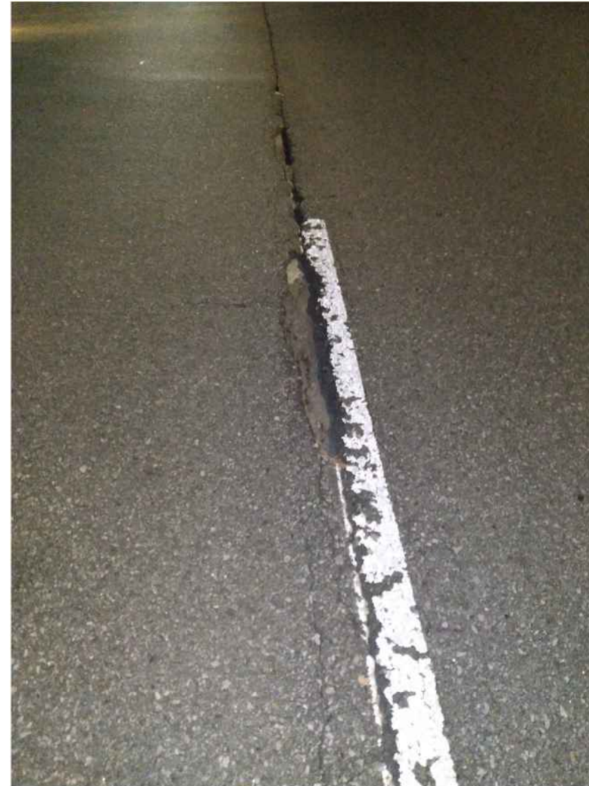
#12: REFLECTIVE CRACKING AT LONGITUDINAL JOINT, SEVERE JOINT DEGRADATION, TYPICAL
