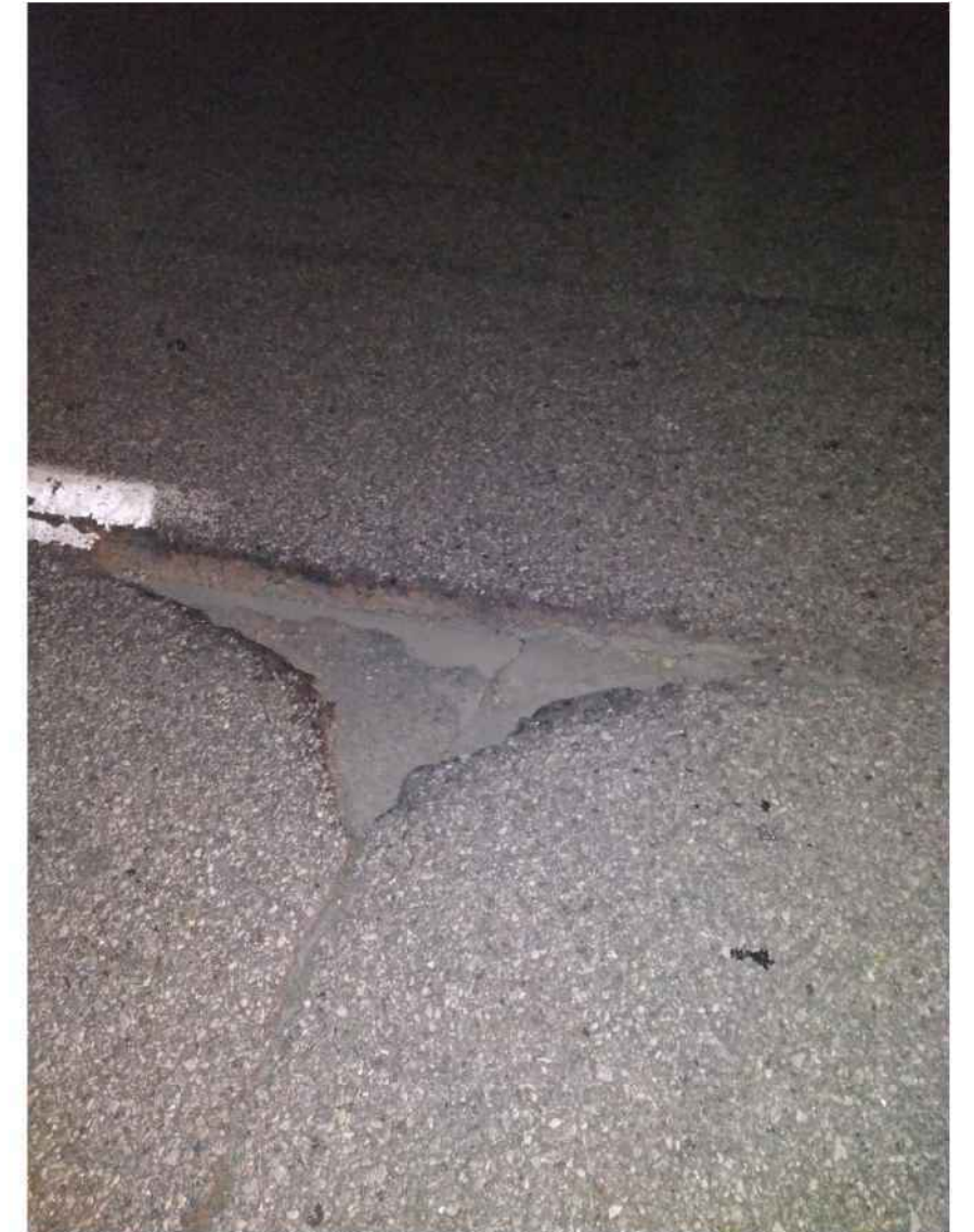
#13: REFLECTIVE CRACKING AT LONGITUDINAL AND TRANSVERSE JOINTS, SEVERE DEGRADATION OF OVERLAY, TYPICAL
