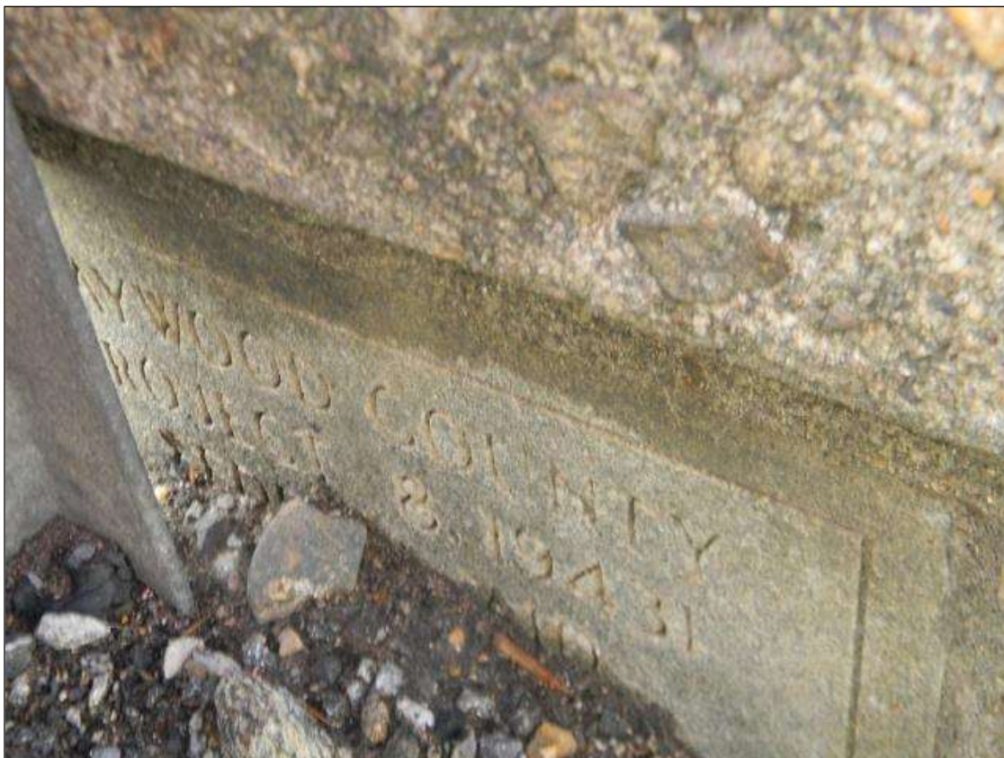
BRIDGE PLATE IS OBSCURED BY THE GUARDRAIL AND DIRT.
