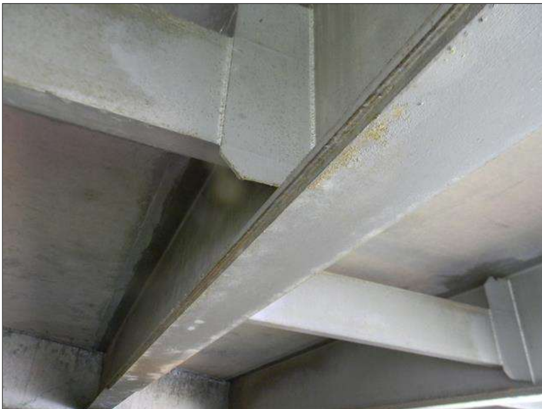
Span 3 Beam 2: FRECKLED RUST ALONG THE BOTTOM FLANGE AND LOWER 2" OF THE WEB.
