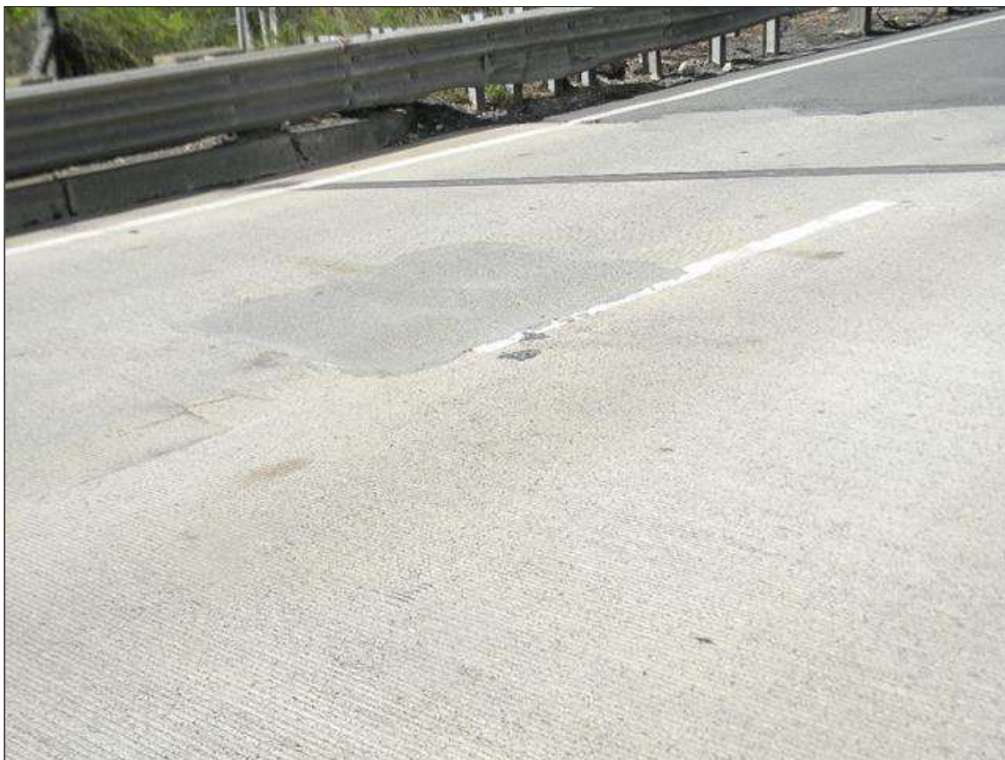
Span 1 Latex Modified Concrete Wearing Surface: RIGHT LANE HAS A 5' WIDE X 6' LONG PATCH IN GOOD CONDITION.
