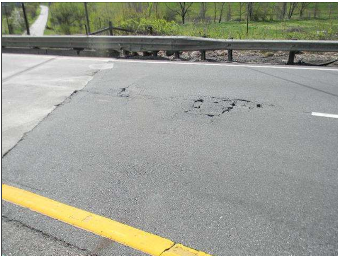
WEST APPROACH ASPHALT WEARING SURFACE IS BREAKING UP IN A 3' WIDE X 9' LONG AREA ALONG THE C/L.
