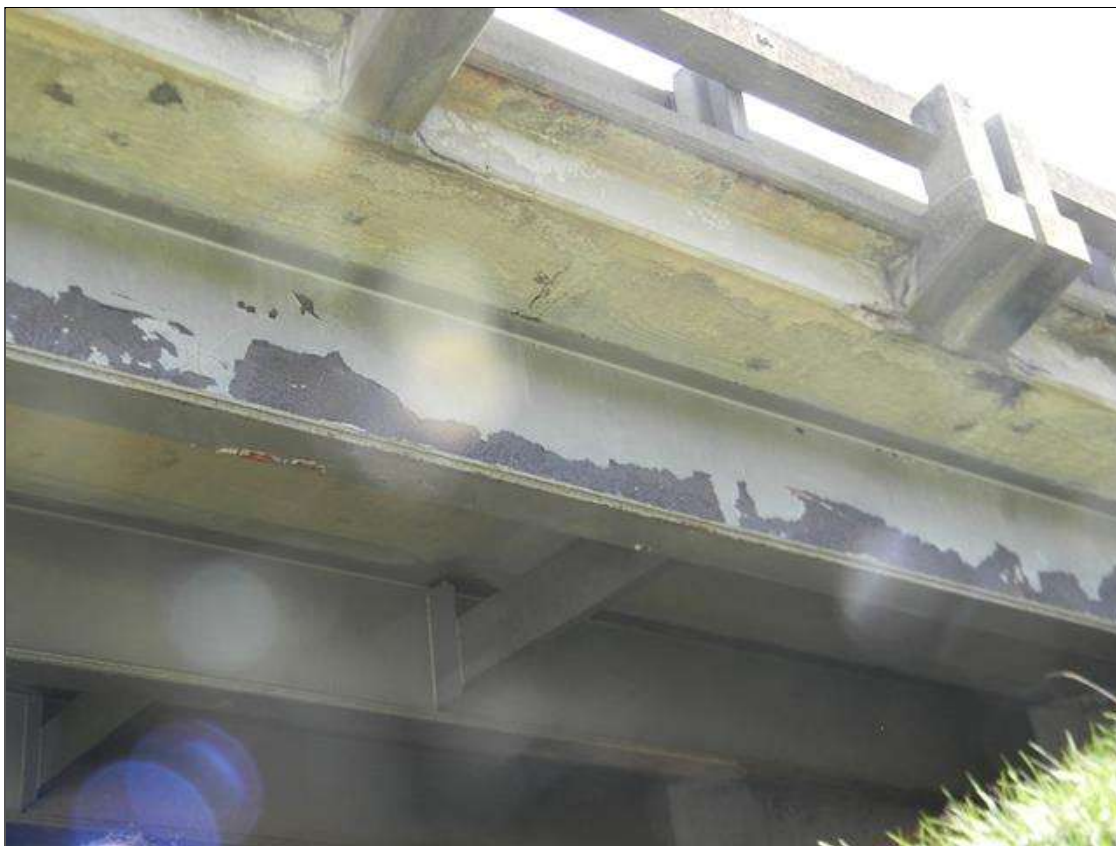
Span 3 Beam 4: PEELING PAINT ALLOWING SURFACE CORROSION ON THE EXTERIOR OF THE WEB.
