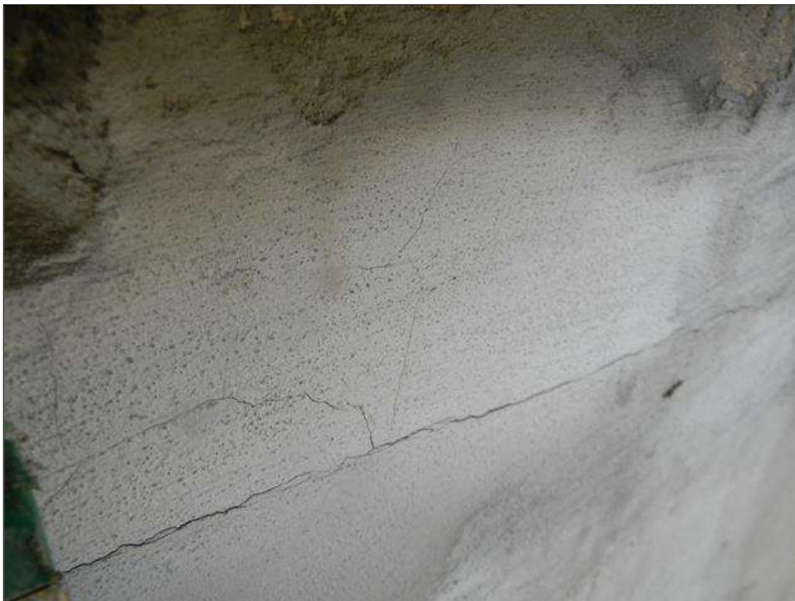
Bent 1 Cap 1: PATCH ON THE EAST FACE UNDER BEAM 1 HAS H/L CRACKING.
