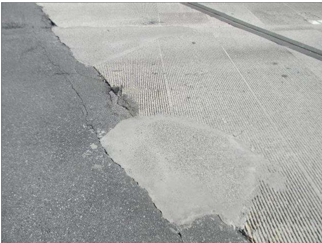
Approach 1: THE EAST APPROACH WEARING SURFACE AND APPROACH SLAB ARE PATCHED IN THE RIGHT LANE. PATCHES ARE IN GOOD CONDITION.
