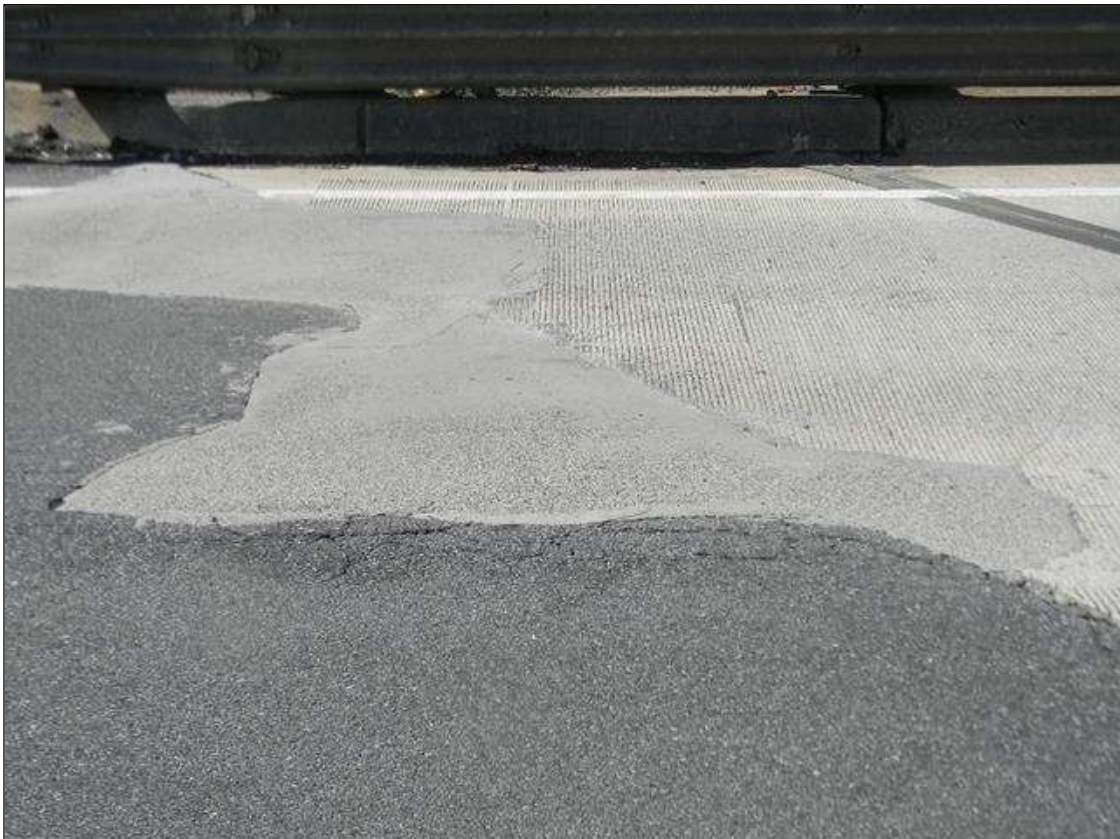
Approach 2: THE EAST APPROACH WEARING SURFACE AND APPROACH SLAB ARE PATCHED IN THE RIGHT LANE. PATCHES ARE IN GOOD CONDITION.
