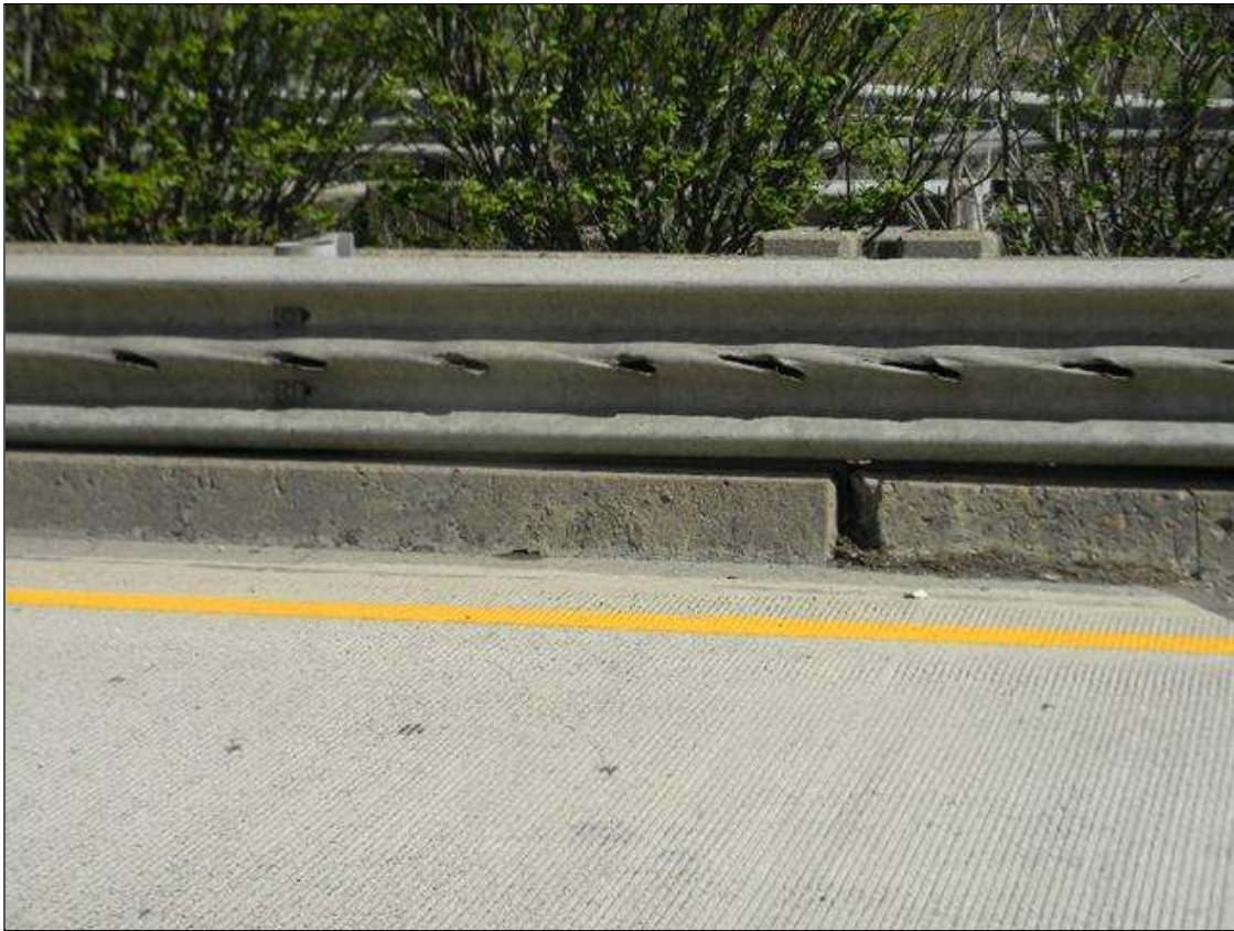
Span 3 Left Bridge Rail: THE LEFT RAIL HAS MINOR SCRAPE DAMAGE, WITH SOME TEARS IN THE STEEL FOR THE FULL LENGTH IN ALL SPANS.
