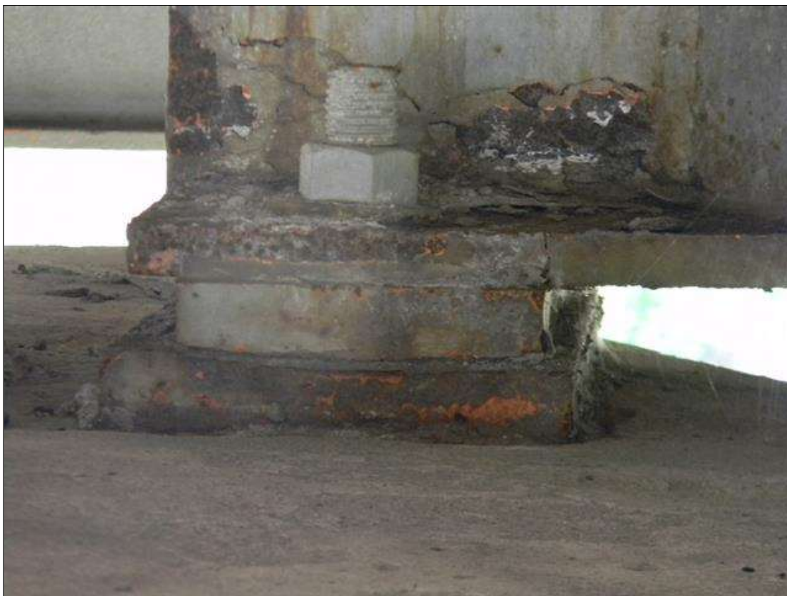
Span 1 Beam 2 Far Bearing: LOSS OF PAINT ALLOWING SURFACE CORROSION ON THE BEARING PLATES.
