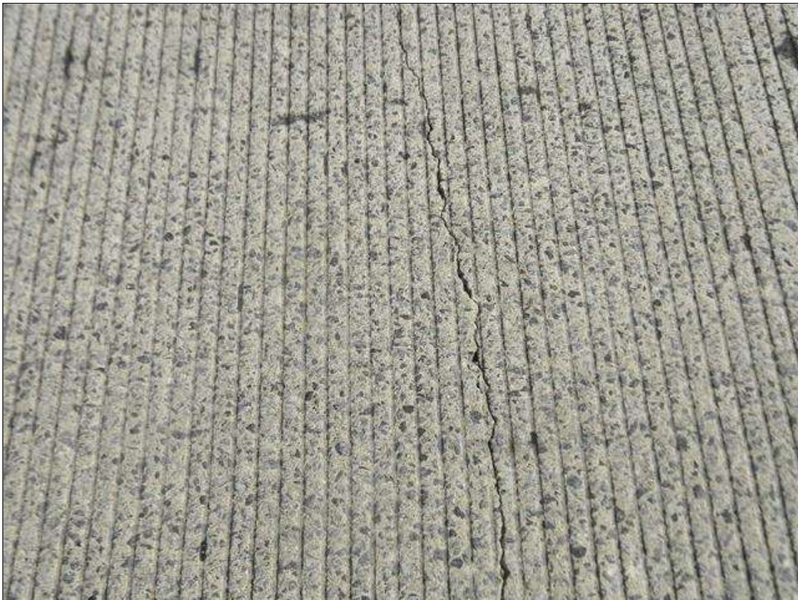
Span 3 Latex Modified Concrete Wearing Surface: WEARING SURFACE HAS SCATTERED MAP CRACKS UP TO 1/16" WIDE.
