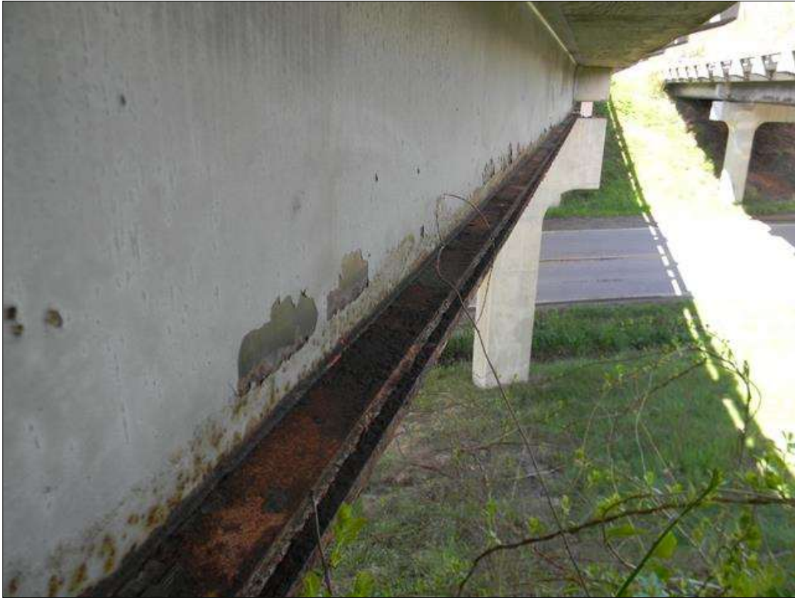
Span 3 Beam 1: LOSS OF PAINT ALONG THE TOP OF THE BOTTOM FLANGE ALLOWING 1/16" PITTING ALONG THE FLANGE AND LOWER WEB.
