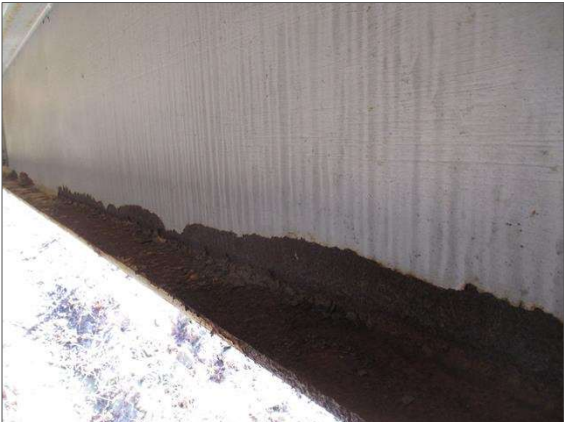
TYPICAL SURFACE CORROSION & DETERIORATED PAINT SYSTEM (SPAN 4, BEAM 6)
