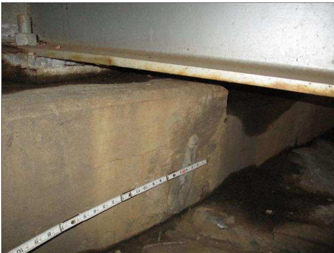
End Bent 1 Abutment: UP TO 0.03" LONGITUDINAL AND MAP CRACKS THROUGHOUT FACE OF CURTAIN WALL IN BAYS 1 THRU 5
