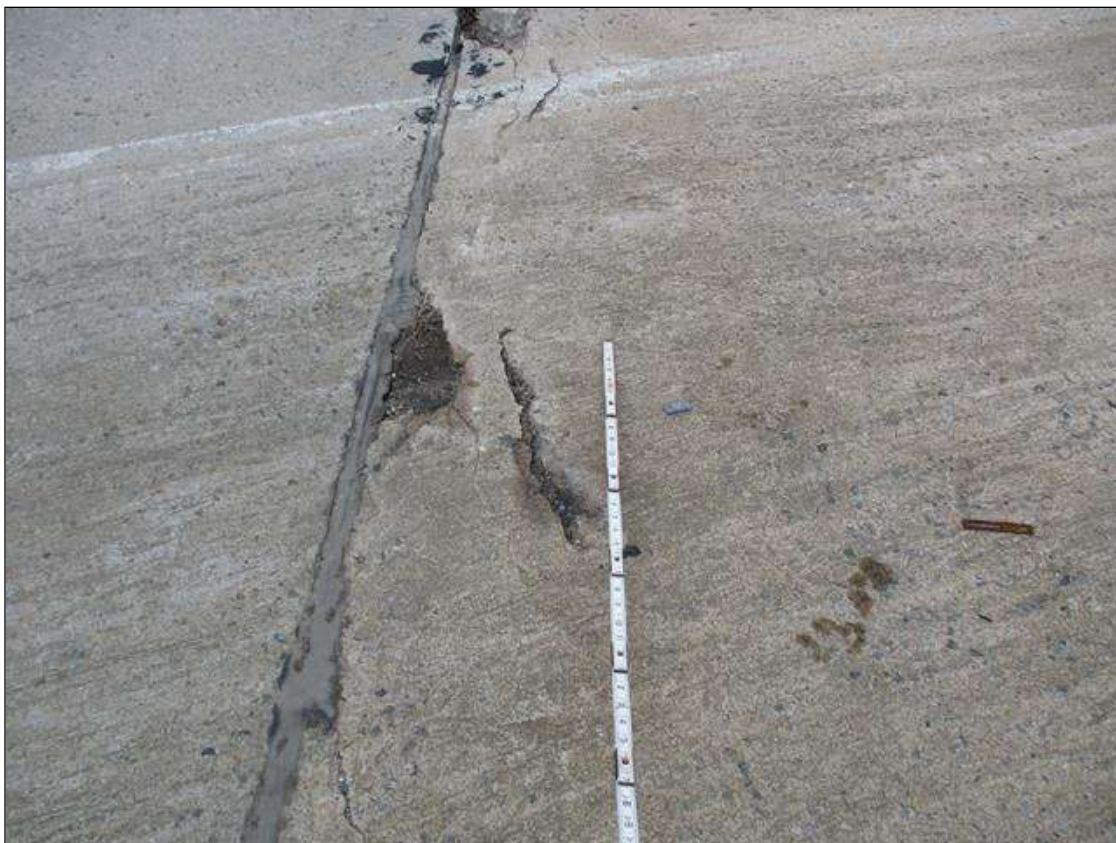
Span 4 Deck: 11" X 4" X 2" DEEP SPALL IN TOP OF DECK IN RIGHT SHOULDER AT BENT 3 JOINT
