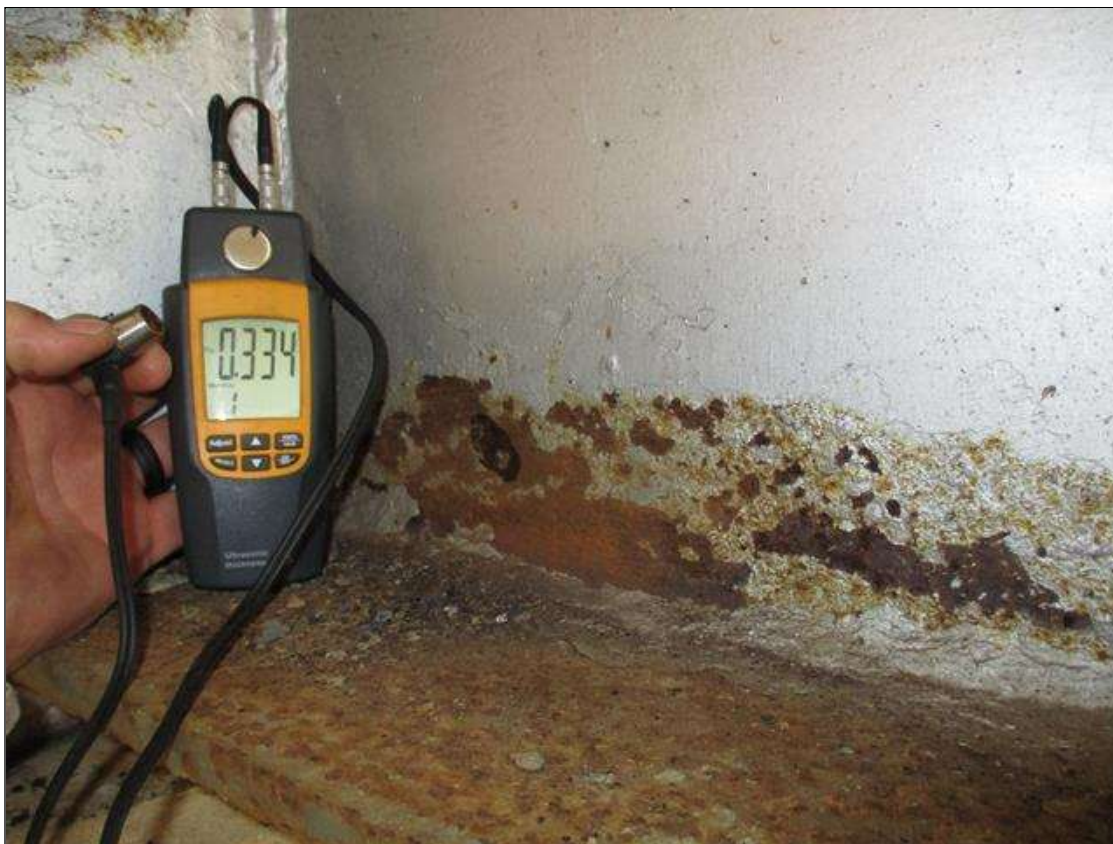
Span 2 Beam 4: (PAR) CORROSION ALONG LEFT FACE OF WEB AND BOTTOM FLANGE UP TO 60" LONG X 5" HIGH WITH DOWN TO 0.334" RESIDUAL WEB, AND 60" LONG X 11 3/4" WIDE DOWN TO 9/16" RESIDUAL FLANGE AT BENT 1 BEARING
