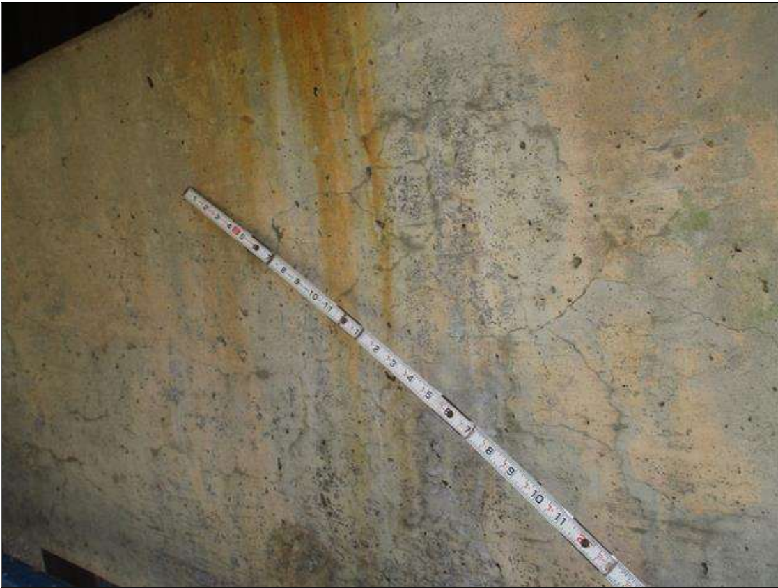
Bent 3 Cap 1: UP TO 1/4" LONGITUDINAL AND HORIZONTAL CRACKS AND HAIRLINE MAP CRACKING WITH AND WITHOUT EFFLORESCENCE IN BOTTOM AND BOTH FACES OF CAP
