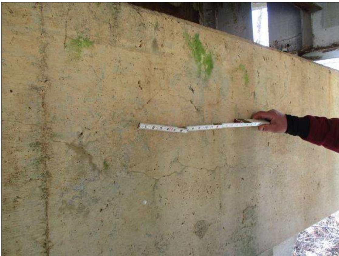
Bent 2 Cap 1: 48" SECTION OF UP TO 1/16" HORIZONTAL AND MAP CRACKS IN SPAN 2 FACE AND BOTTOM OF CAP, APPROXIMATELY 6' TO LEFT OF COLUMN 2
