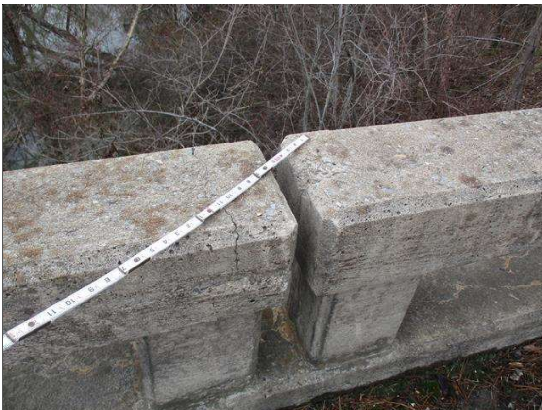
Span 1 Right Bridge Rail: 3 1/2" X 3" X 1" DEEP SPALL IN TOP OF RAIL, APPROXIMATELY 18' FROM BENT 1 JOINT
