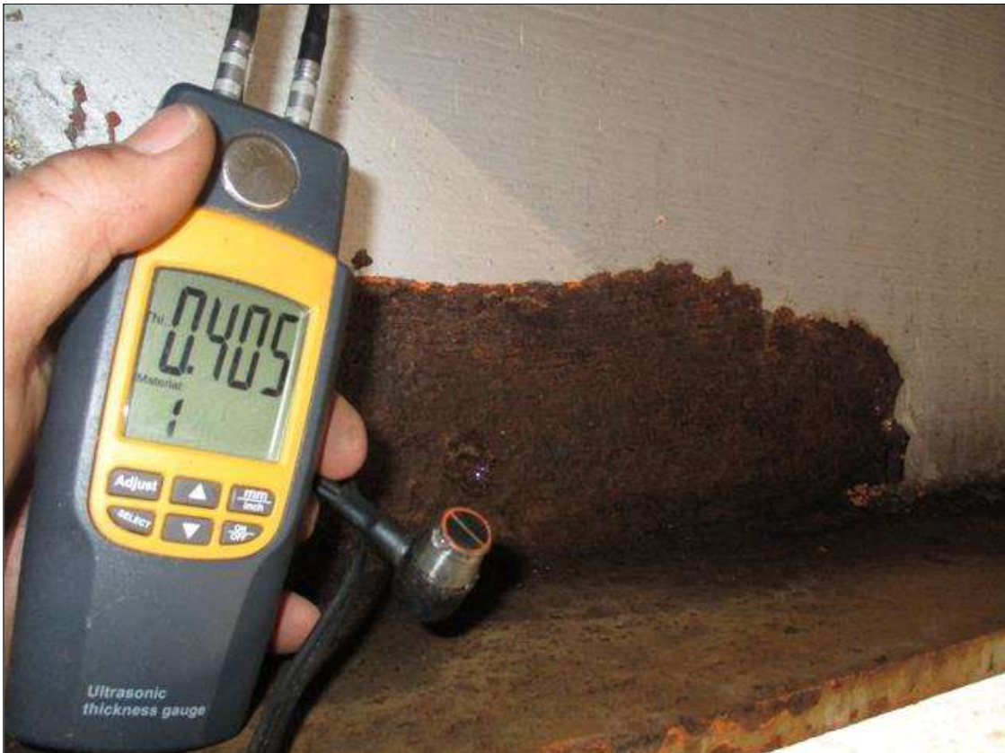
Span 3 Beam 2: (PAR) CORROSION ALONG BOTH FACES OF WEB UP TO 12" LONG X 24" HIGH DOWN TO 0.405" RESIDUAL WEB AT END OF BEAM AT BENT 2
