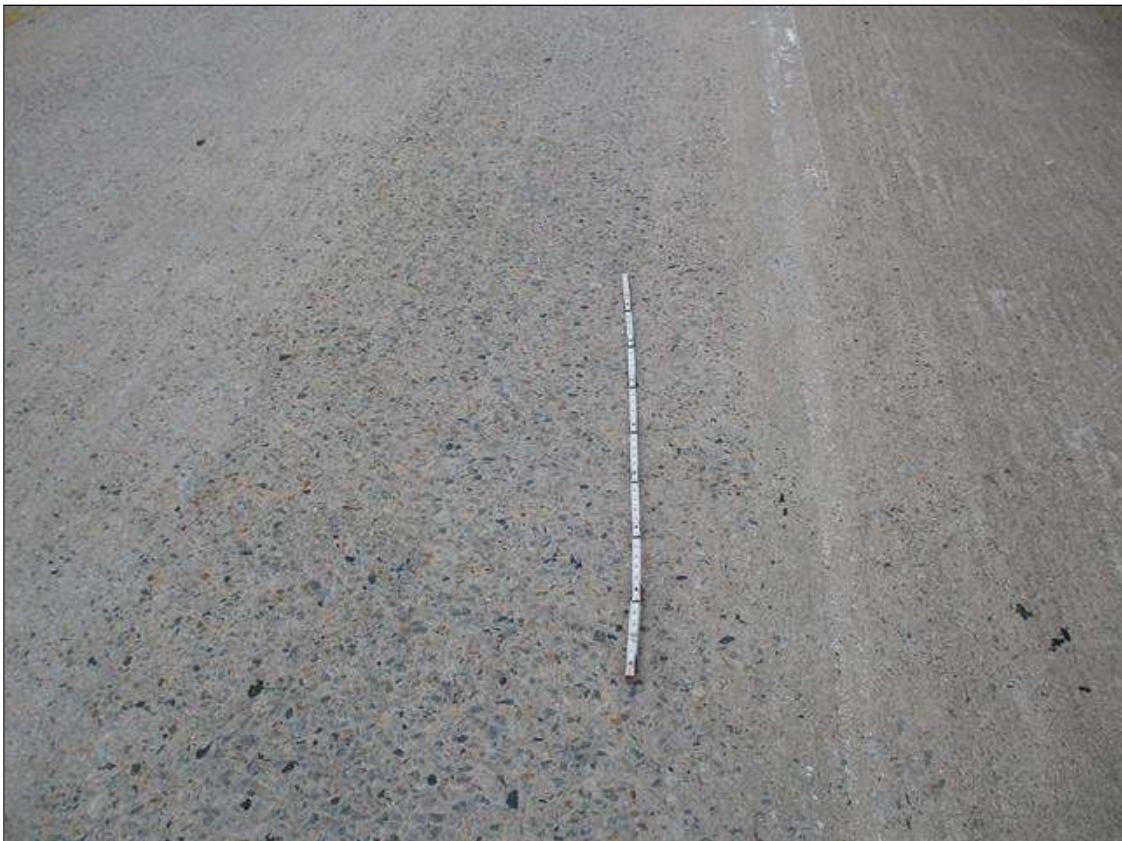
Span 1 Deck: 1320 SQUARE FEET OF SCALING WITH EXPOSED AGGREGATE IN TOP OF DECK THROUGHOUT TRAVEL LANES
