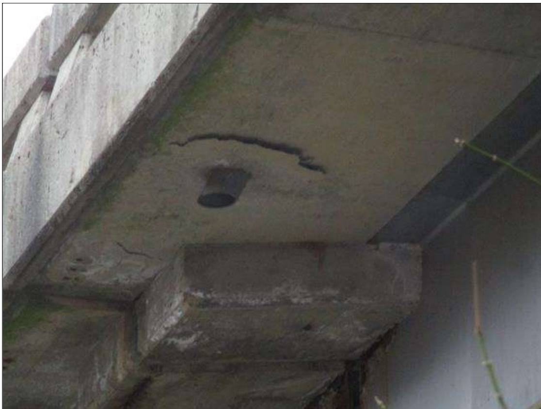
Span 1 Deck: UNDERSIDE, 12" X 11" AREA OF DELAMINATION IN BOTTOM OF LEFT OVERHANG ABOVE BENT 1
