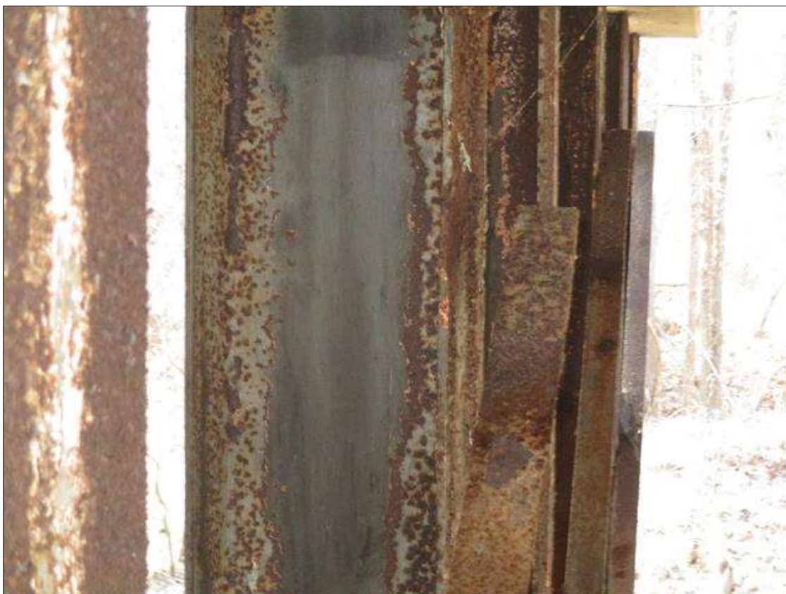
(PAR) AREAS OF 100% SECTION LOSS UP 17" X 3" AND BROKEN AND DETACHED CROSS BRACING INTERMITTENT THROUGHOUT BENT 3
