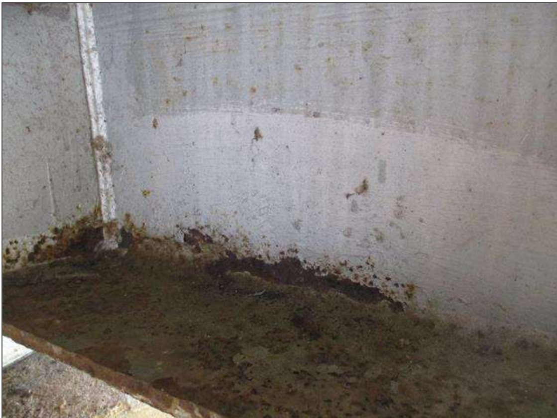
TYPICAL DETERIORATED PAINT SYSTEM (SPAN 2, BEAM 6)
