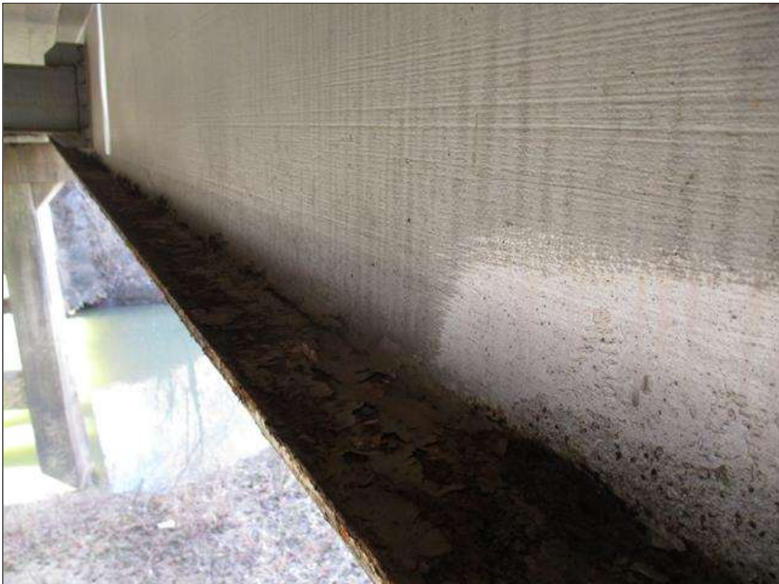
TYPICAL DETERIORATED PAINT SYSTEM (SPAN 3, BEAM 1)
