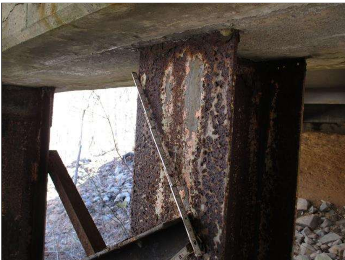
TYPICAL SURFACE CORROSION & DETERIORATED PAINT SYSTEM (BENT 3, PILE 4)
