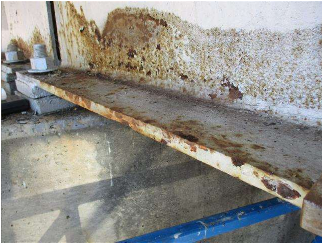
TYPICAL SURFACE OF CORROSION & DETERIORATED PAINT SYSTEM (SPAN 2, BEAM 6)
