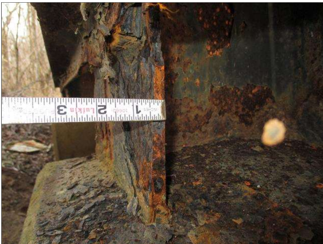
Bent 3 Pile 3: (PAR) CORROSION ALONG BOTH FLANGES UP TO 17" HIGH X 12" WIDE DOWN TO 3/8" RESIDUAL FLANGE ABOVE CONCRETE ENCASEMENT
