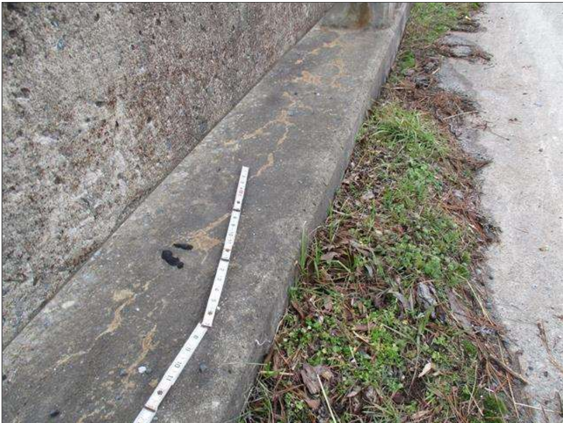
Span 2 Right Bridge Rail: ON TOP OF CURB THROUGHOUT, LESS THAN 0.01" WIDE CRACKING WITH EFFLORESCENCE
