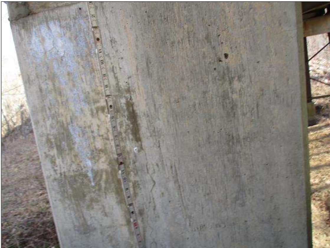
Bent 2 Pile 1: UP TO 0.02" VERTICAL CRACKS AND HAIRLINE MAP CRACKS WITH AND WITHOUT EFFLORESCENCE THROUGHOUT COLUMN
