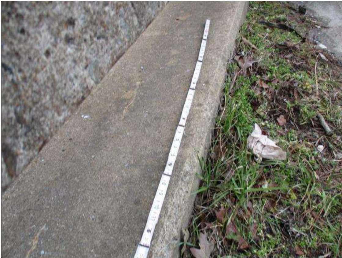
Span 4 Right Bridge Rail: ON TOP OF CURB THROUGHOUT, LESS THAN 0.01" WIDE CRACKING WITH EFFLORESCENCE
