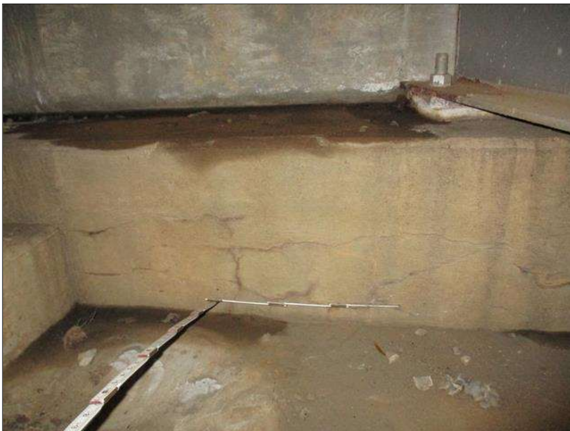
End Bent 1 Abutment: UP TO 0.03" LONGITUDINAL AND MAP CRACKS THROUGHOUT FACE OF CURTAIN WALL IN BAYS 1 THRU 5
