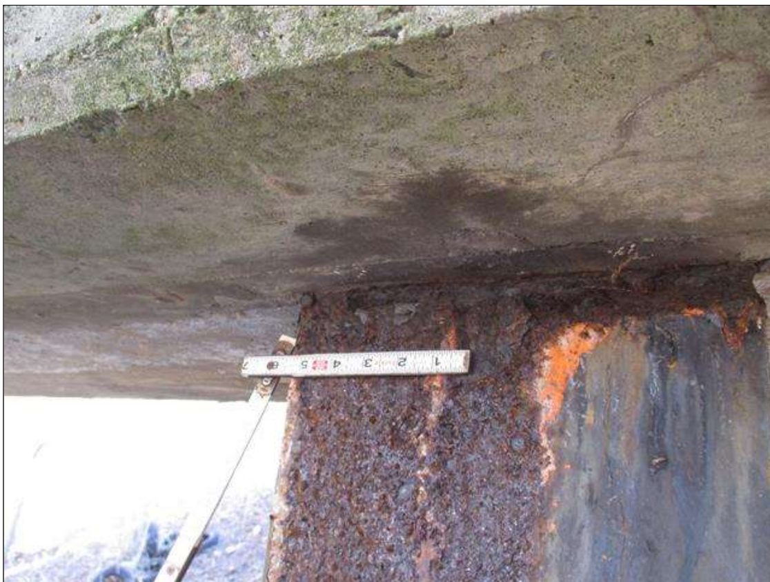
Bent 3 Pile 2: (PAR) CORROSION ALONG NEAR FLANGE UP TO 3" HIGH X 12" WIDE DOWN TO 1/4" RESIDUAL FLANGE WITH 3/16" DIAMETER HOLE AT BOTTOM OF CAP UP TO 3" LONG
