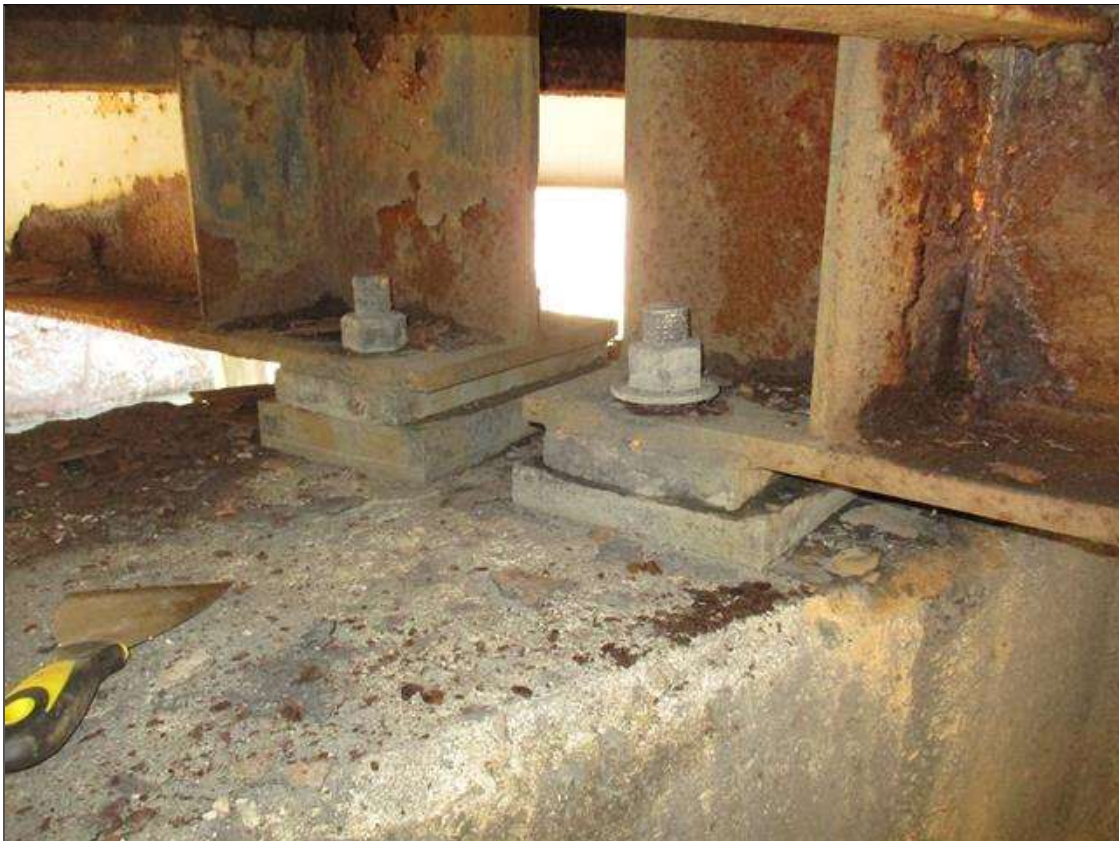
Span 4 Beam 4 - Far Bearing - Protective System: DETERIORATED PAINT SYSTEM THROUGHOUT BEAM 4 BEARING
