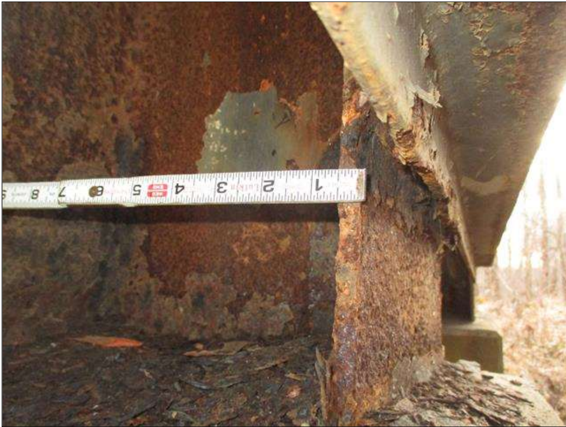
Bent 3 Pile 9: (PAR) CORROSION ALONG BOTH FLANGES UP TO 12" HIGH X 12" WIDE DOWN TO 5/16" RESIDUAL FLANGE ABOVE CONCRETE ENCASEMENT
