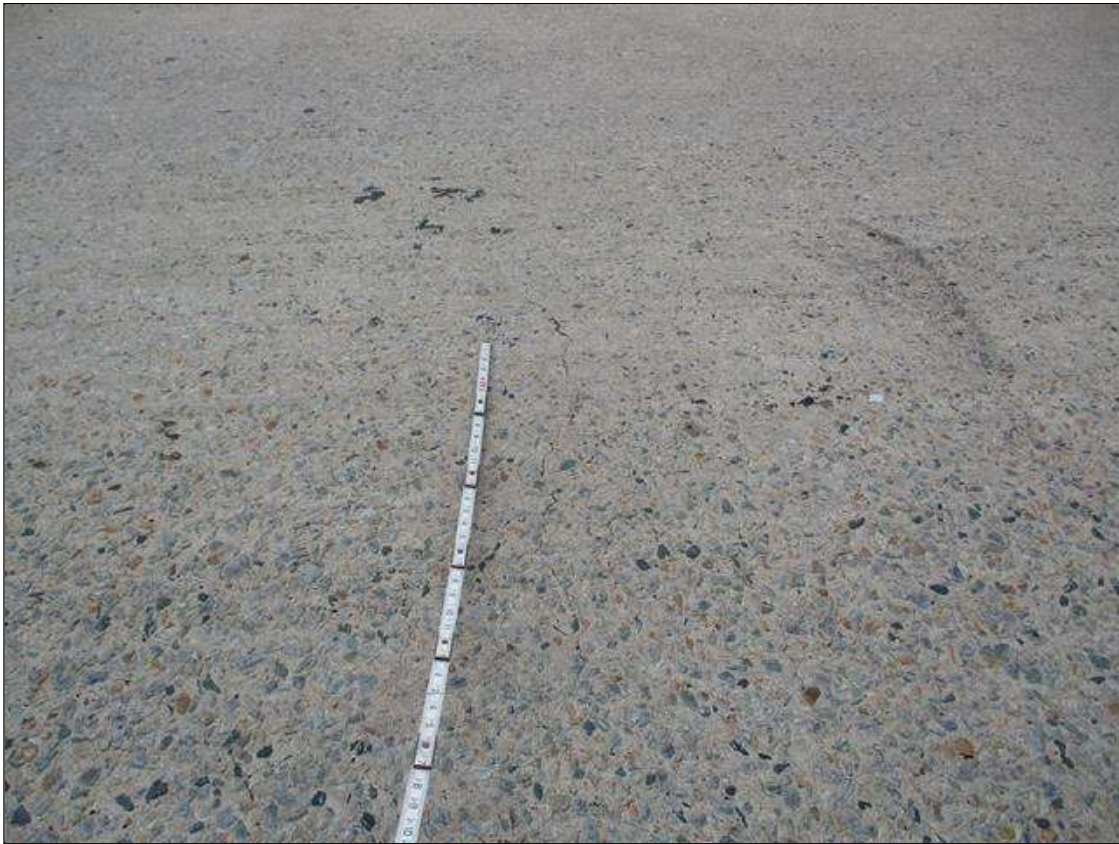
Span 1 Deck: UP TO 0.035" TRANSVERSE CRACKS IN TOP OF DECK IN TRAVEL LANES WITHIN 3' OF END BENT 1 FILL FACE
