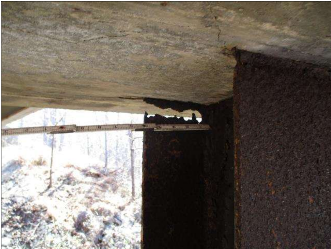
Bent 3 Pile 9: (PAR) CORROSION ALONG BOTH FLANGES UP TO 20" HIGH X 12" WIDE, 100% SECTION LOSS ON FLANGE WITH UP TO 4" WIDE X 1 1/2" HIGH LOSS OF SECTIONS AT BOTTOM OF CAP
