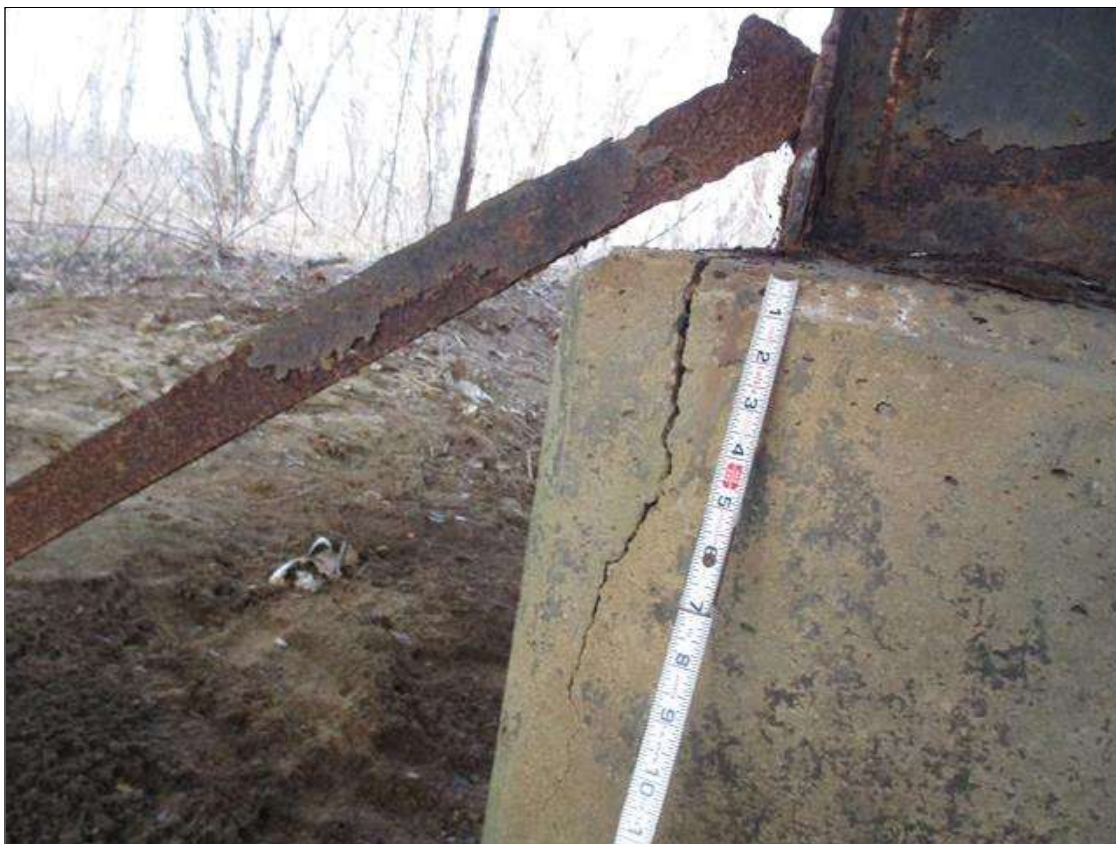
UP TO 1/8" TRANSVERSE & VERTICAL CRACKS IN ENCASEMENT (BENT 3, PILE 5)
