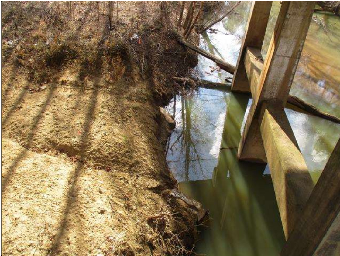
SLUMPING ALONG ALL BANKS
