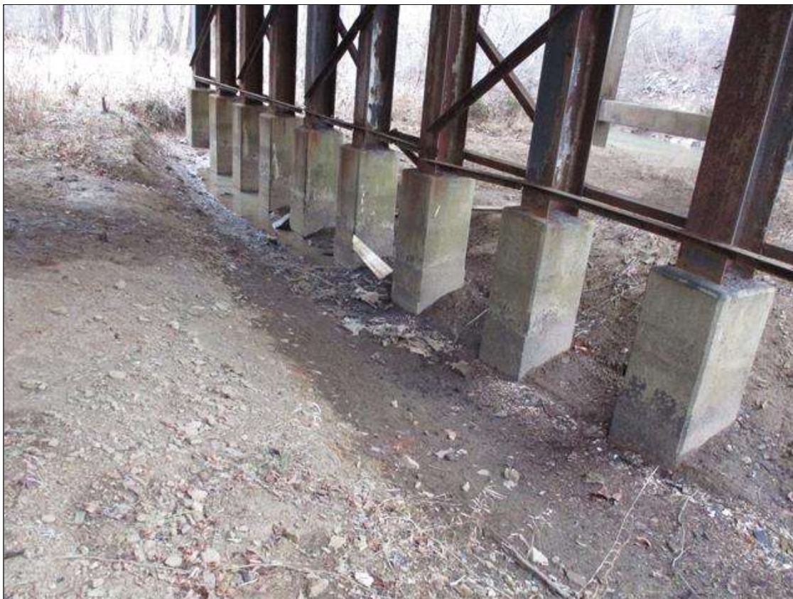
AT BENT 3, SCOUR HOLE AROUND ALL PILES, 50' LONG X 12' WIDE X UP TO 2.5' DEEP
