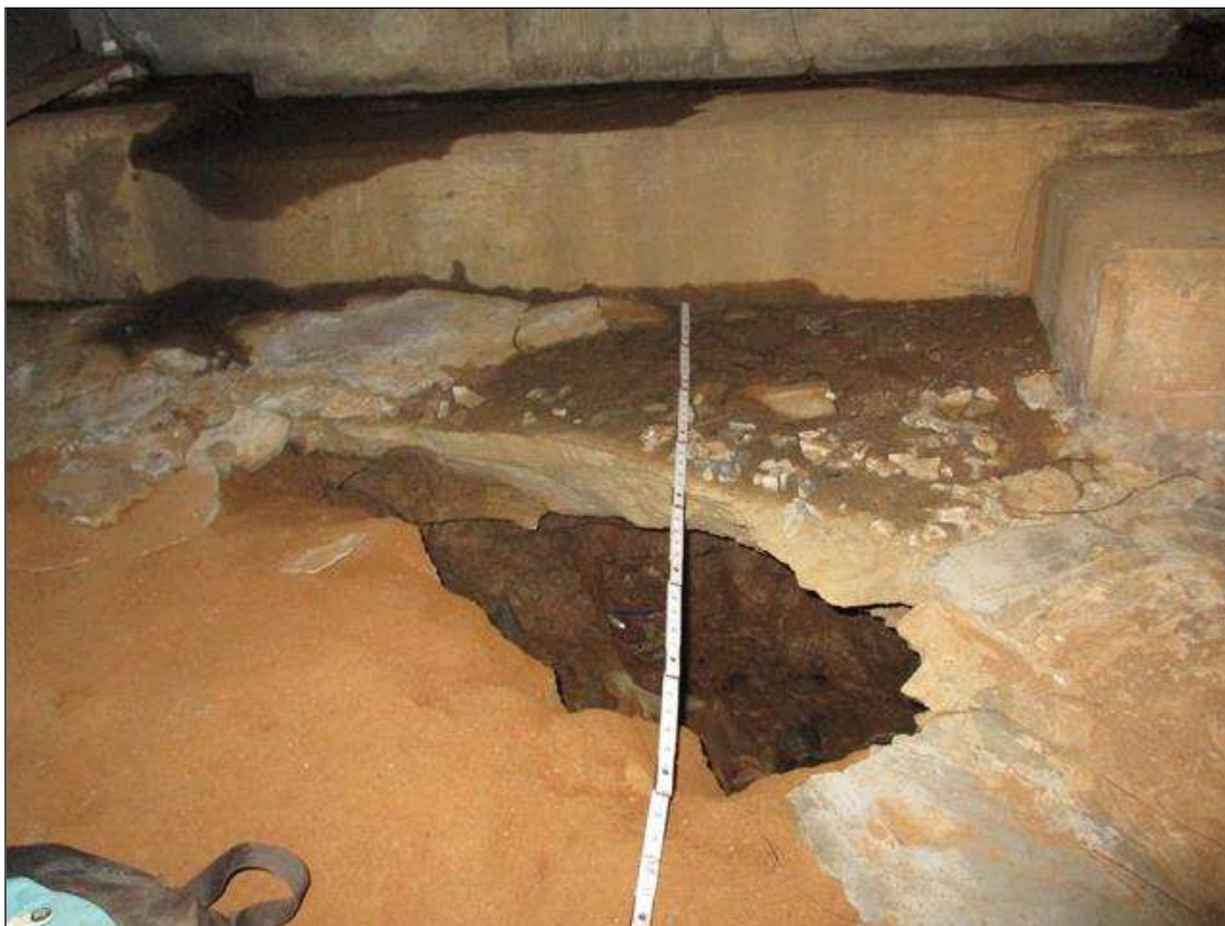
(PAR) SLOPE @ END BENT HAS EROSION AREA 5'x 8'x 4' DEEP UNDERMINING CAP BETWEEN BEAMS 1 & 2
