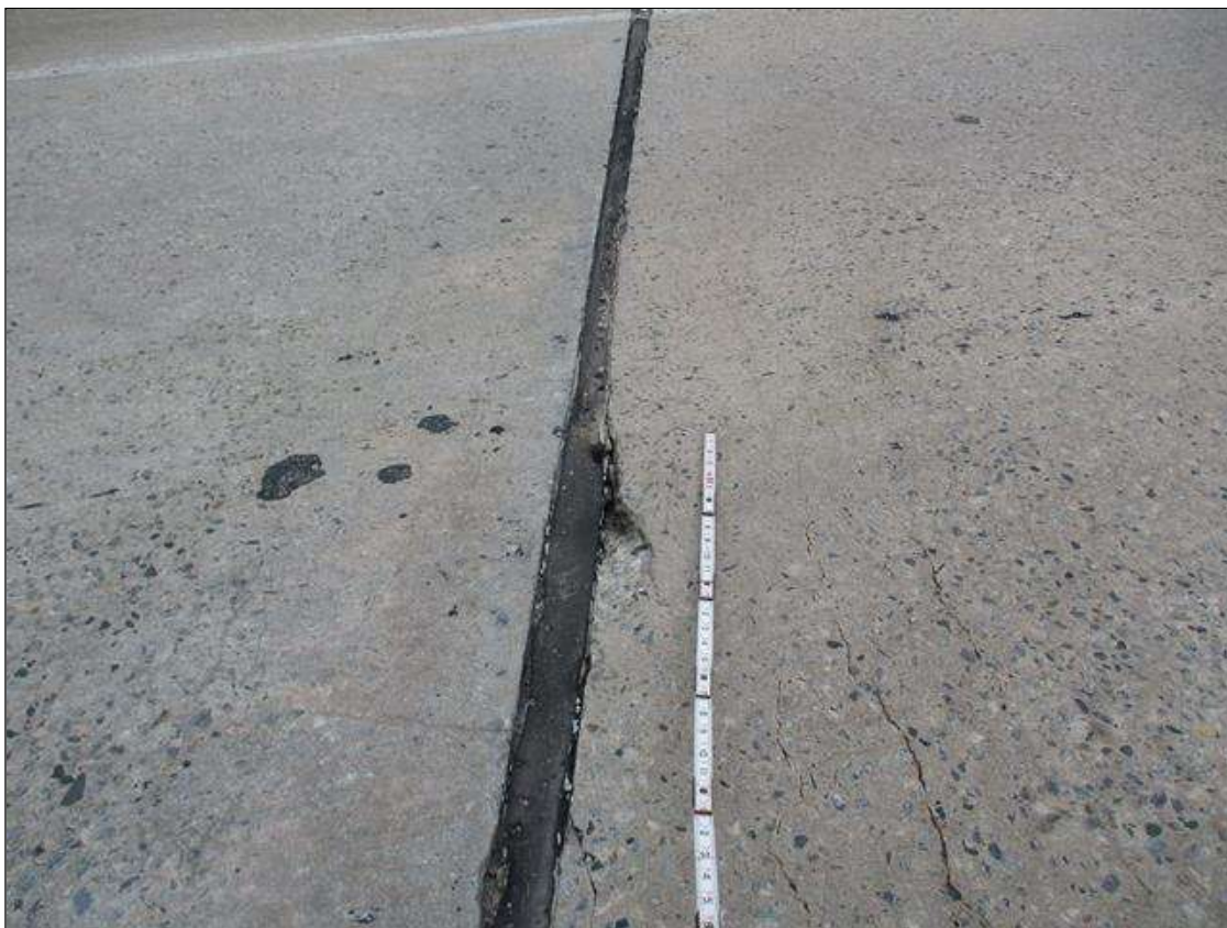
Span 2 Deck: UP TO 0.04" TRANSVERSE CRACKS IN TOP OF DECK IN TRAVEL LANES AT BENT 2 JOINT
