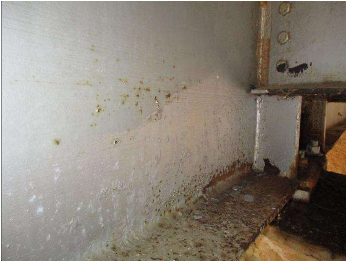
Span 3 Beam 3 - Protective System: DETERIORATED PAINT SYSTEM ALONG BOTH FACES OF WEB AND BOTTOM FLANGE UP TO 15" LONG X 5" HIGH IN WEB, AND 18" LONG X 11 3/4" WIDE IN FLANGE AT BENT 3 BEARING
