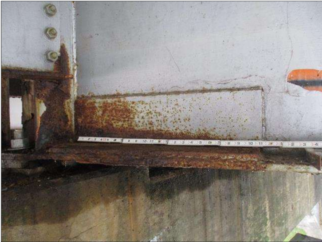
Span 2 Beam 3: SURFACE CORROSION THROUGHOUT 24" LONG X 5" WIDE X 6" HIGH PLATE REPAIR WELDED TO RIGHT FACE OF WEB AND BOTTOM FLANGE AT BENT 1 ON BOTH SIDES
