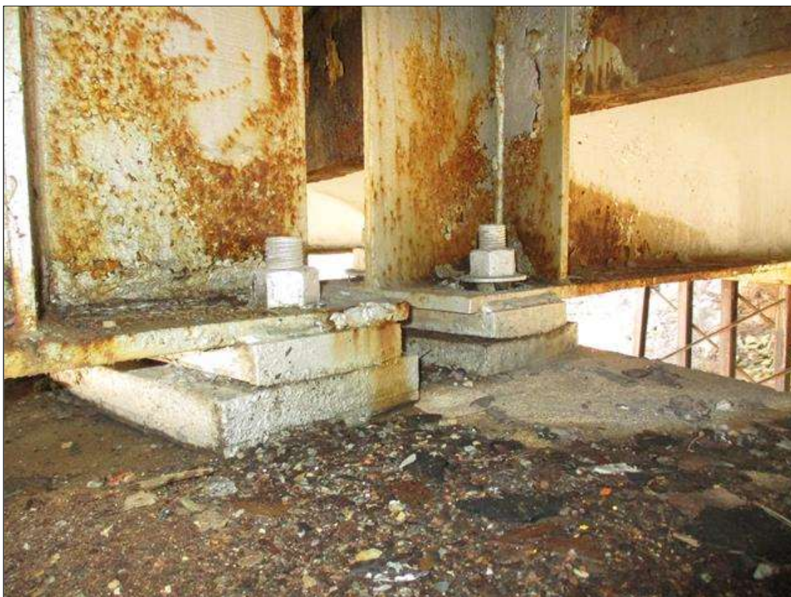
Span 2 Beam 4 - Near Bearing - Protective System: AREAS OF DETERIORATED PAINT SYSTEM THROUGHOUT BEAM 4 BEARING
