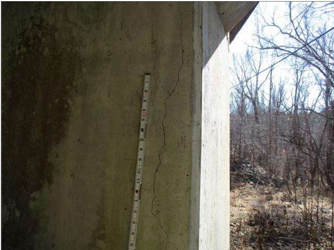
Bent 2 Pile 3: UP TO 8' X 1/16" VERTICAL CRACKS THROUGHOUT COLUMN AT WATER SURFACE & UP TO CAP
