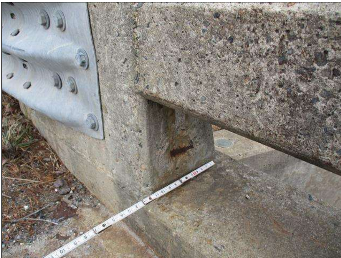
Span 1 Left Bridge Rail: 5" X 3" X 1/2" DEEP SPALL WITH EXPOSED REBAR IN EAST FACE OF END POST, APPROXIMATELY 3' FROM END BENT 1 FILL FACE
