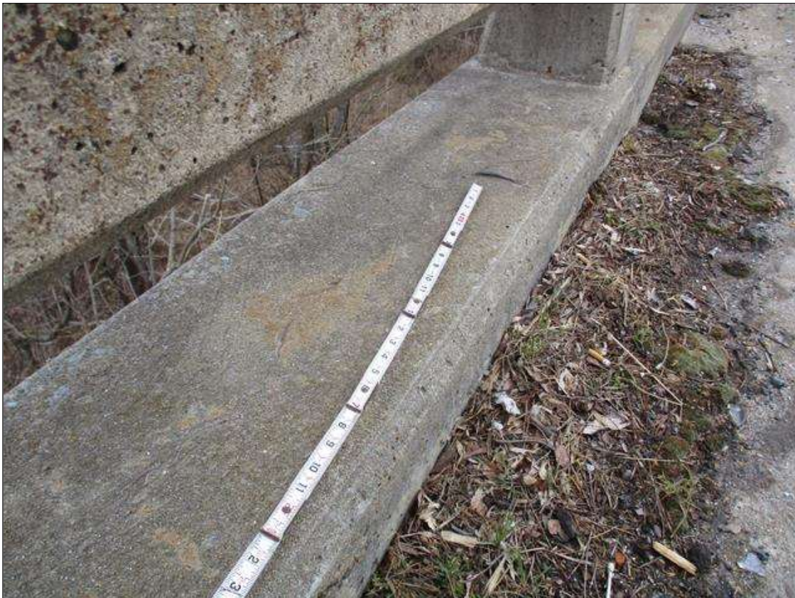
Span 3 Left Bridge Rail: ON TOP OF CURB THROUGHOUT, LESS THAN 0.01" WIDE CRACKING WITH EFFLORESCENCE
