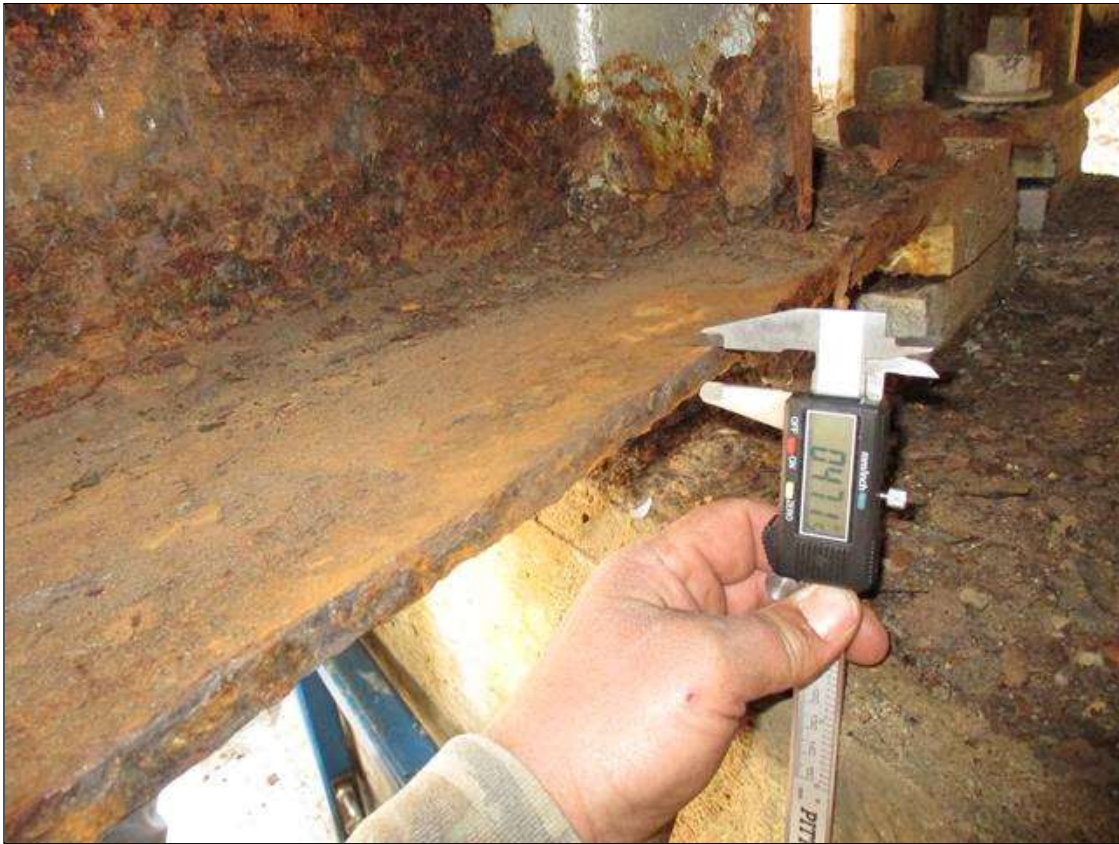
Span 3 Beam 1: (PAR) CORROSION ALONG RIGHT FACE OF WEB AND BOTTOM FLANGE UP TO 34" LONG X 5" HIGH DOWN TO 0.470" RESIDUAL WEB, AND 36" LONG X 5" WIDE DOWN TO 0.401" RESIDUAL FLANGE AT BENT 3 BEARING
