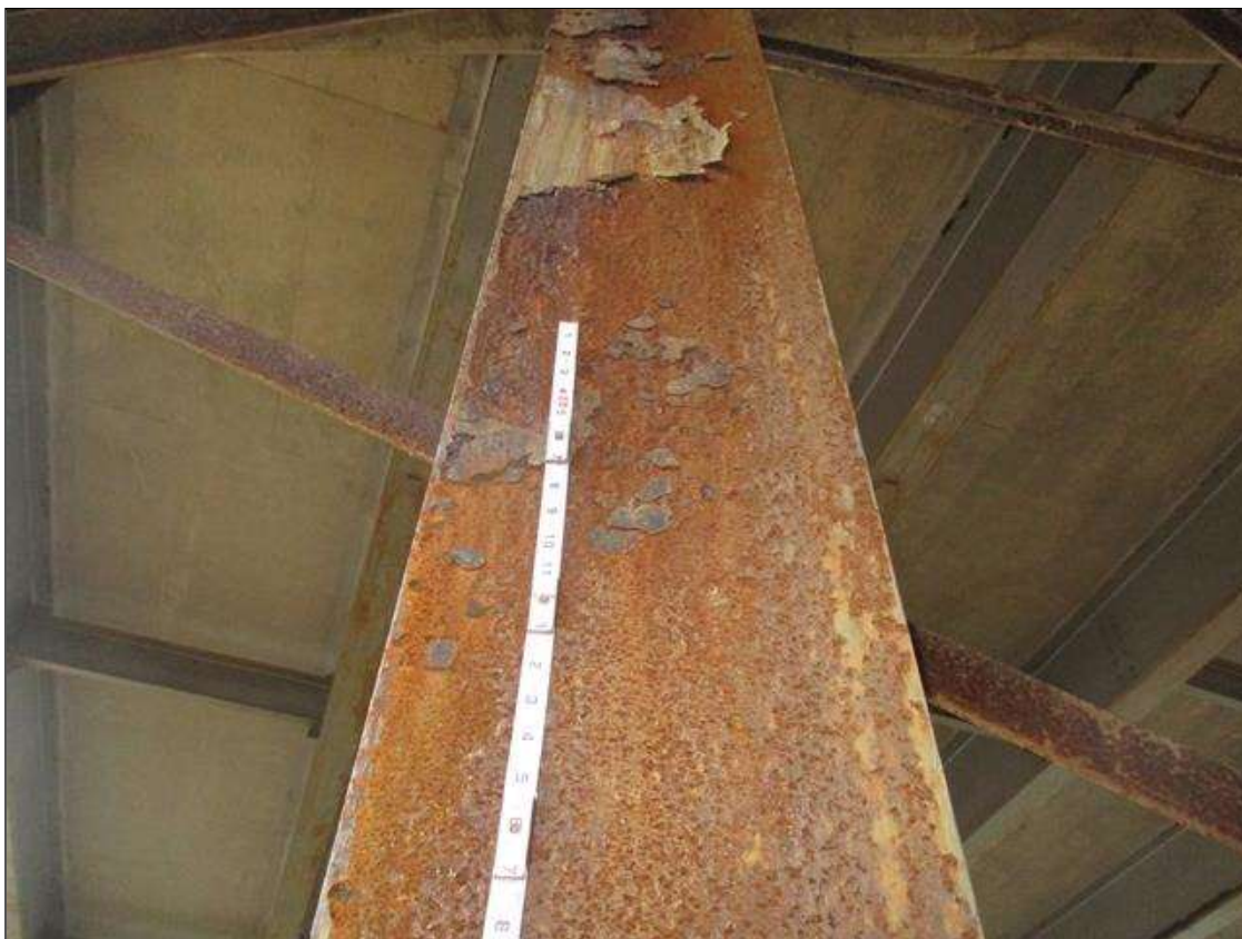
TYPICAL SURFACE CORROSION & DETERIORATED PAINT SYSTEM (BENT 3, PILE 8)
