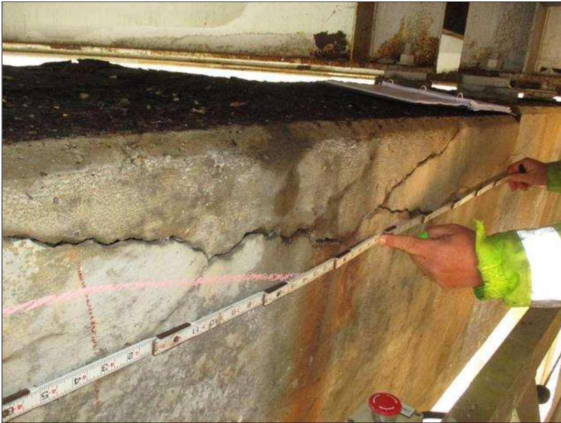
Bent 1 Cap 1: BOTH FACES, UP TO 1/4" LONGITUDINAL AND HORIZONTAL CRACKS AND HAIRLINE MAP CRACKS WITH AND WITHOUT EFFLORESCENCE AND RUST STAINING WITH UP TO 8' X 31" AREAS OF DELAMINATION THROUGHOUT CAP BENEATH BAYS 2 THRU 4
