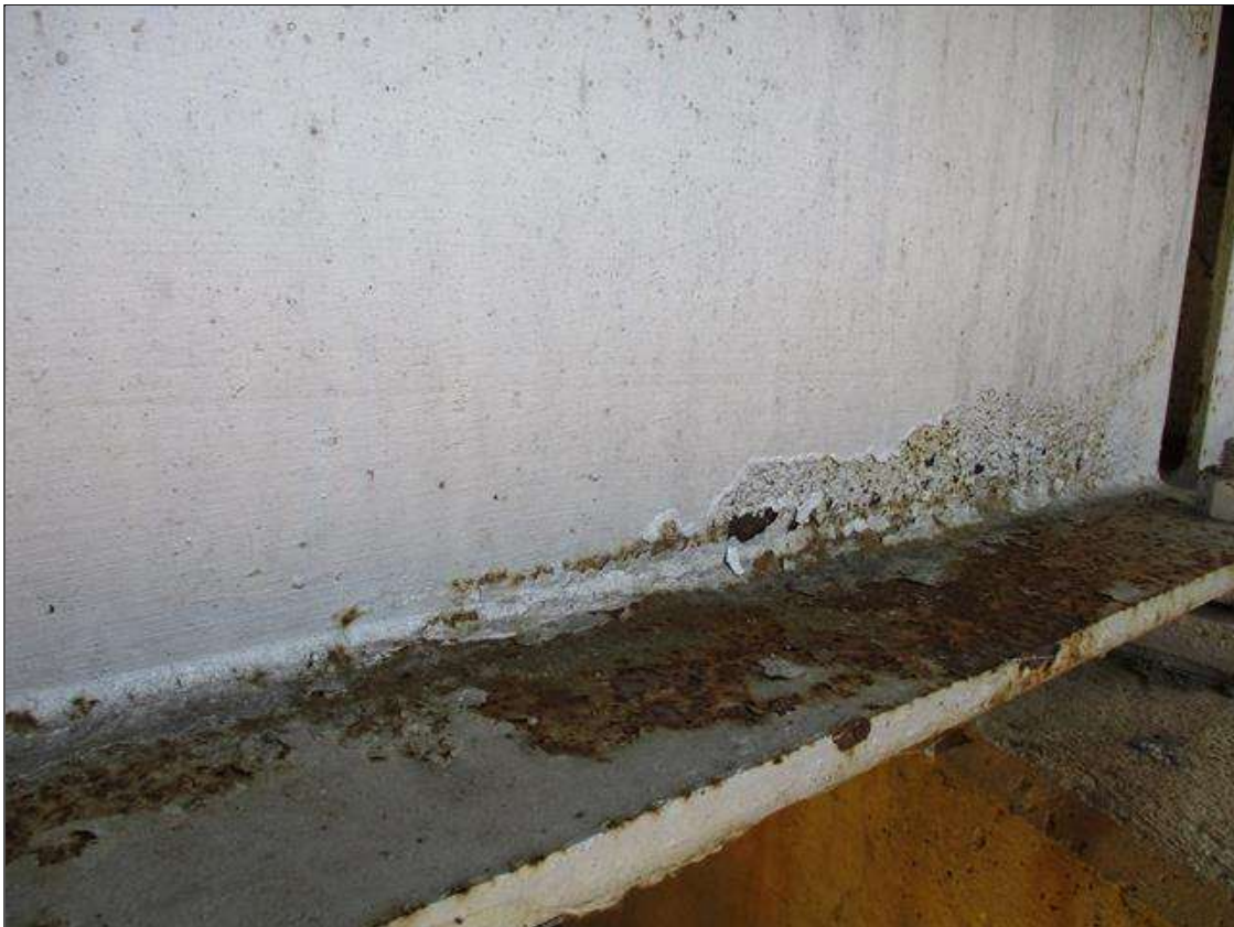
TYPICAL SURFACE CORROSION & DETERIORATED PAINT SYSTEM (SPAN 2, BEAM 5)
