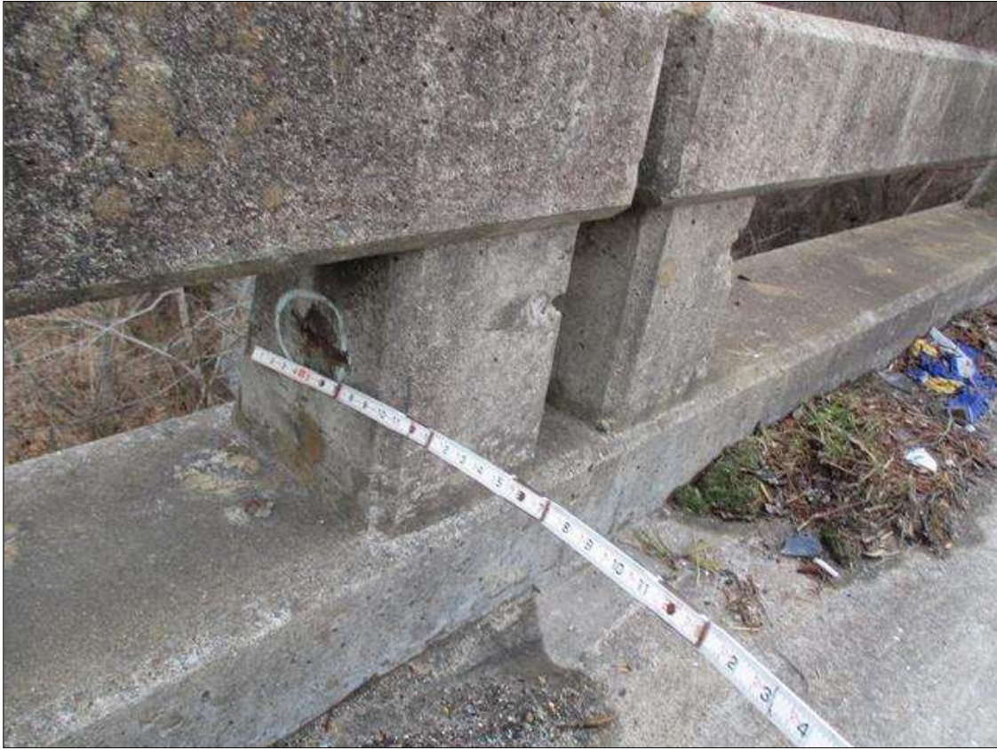
Span 3 Right Bridge Rail: THREE (3) SPALLS UP TO 4" X 3 1/2" X 1/4" DEEP IN FACE OF RAIL AND RAIL POSTS IN VARIOUS LOCATIONS
