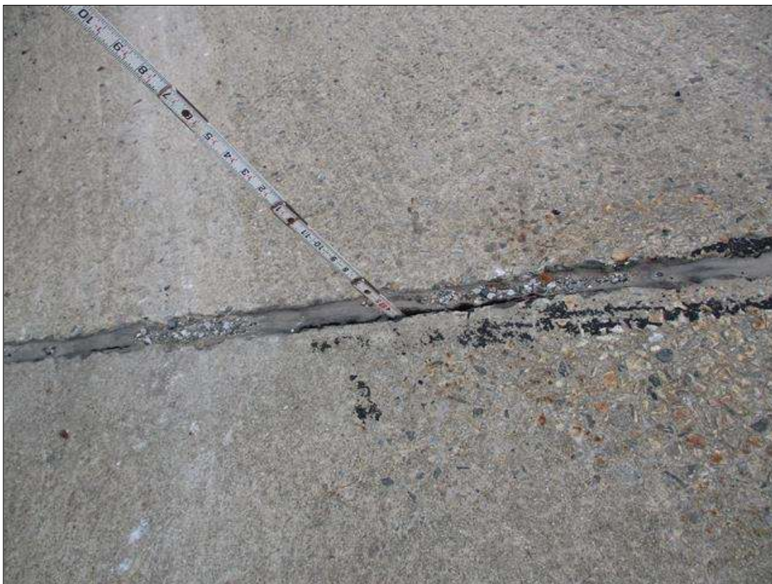
FULL DEPTH SEPARATION OF JOINT MATERIAL IN VARIOUS LOCATIONS (TYPICAL OF ALL JOINTS)
