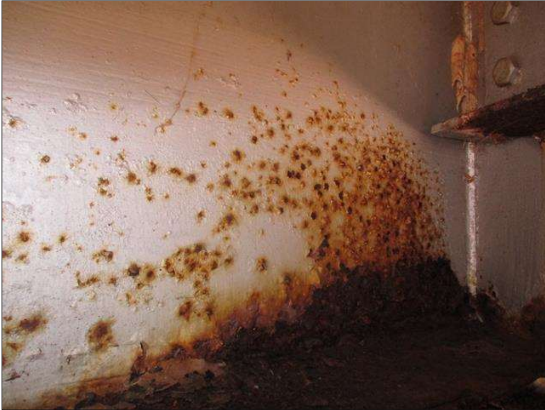
Span 2 Beam 3 - Protective System: DETERIORATED PAINT SYSTEM ALONG BOTH FACES OF WEB AND BOTTOM FLANGE UP TO 25" LONG X 24" HIGH IN WEB, AND 24" LONG X 11 3/4" WIDE IN FLANGE AT BENT 2 BEARING
