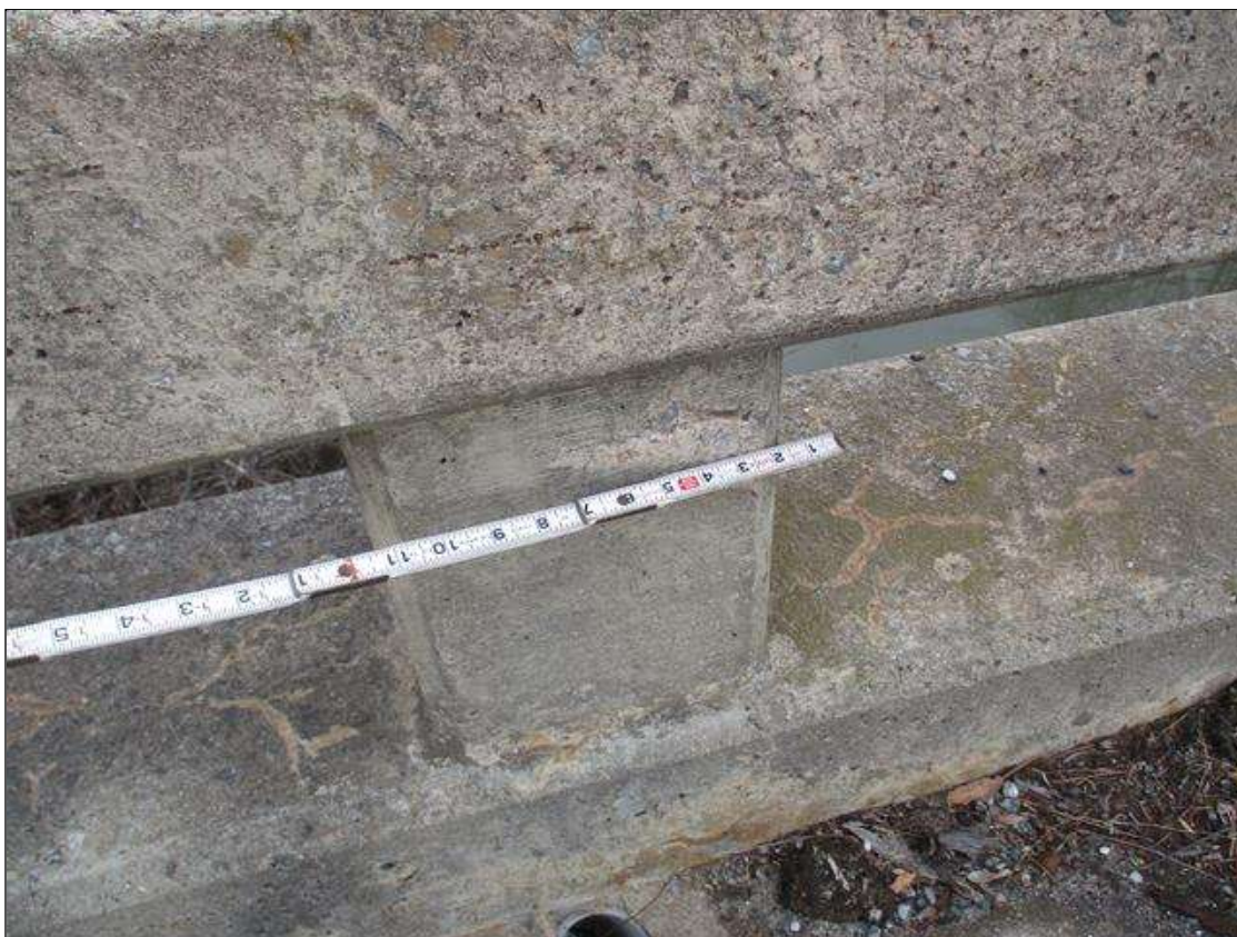
Span 2 Left Bridge Rail: FIVE (5) SPALLS UP TO 5" X 3 1/2" X 1/4" DEEP IN FACE OF RAIL POSTS IN VARIOUS LOCATIONS
