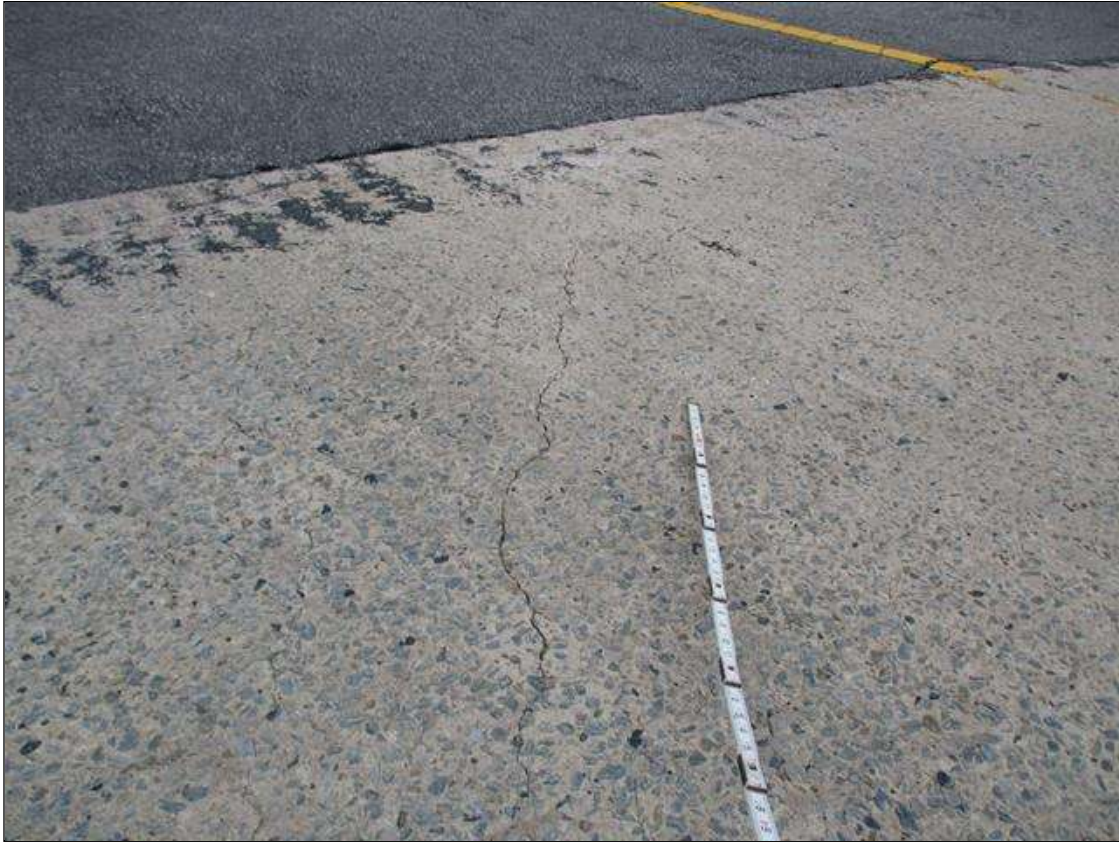
Span 4 Deck: 58" X UP TO 1/8" DIAGONAL CRACK IN TOP OF DECK IN WESTBOUND LANE NEAR END BENT 2 FILL FACE
