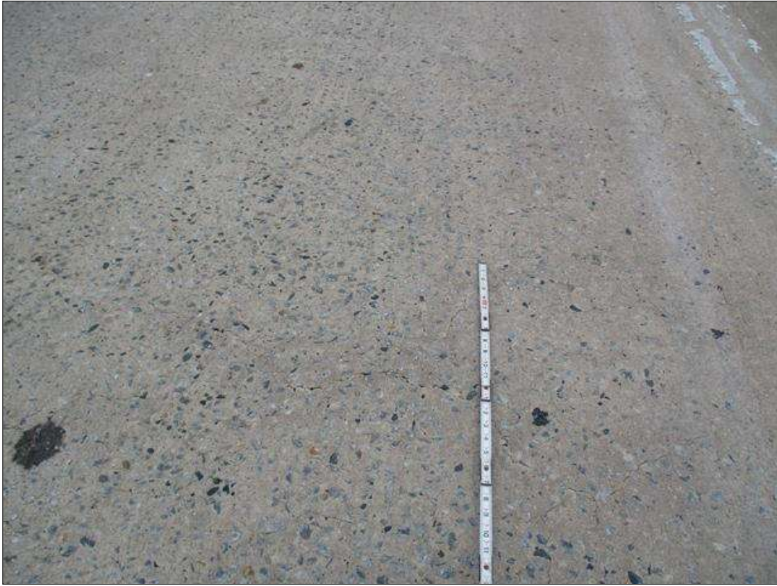
Span 2 Deck: UP TO 0.02" MAP CRACKS IN TOP OF DECK IN VARIOUS LOCATIONS
