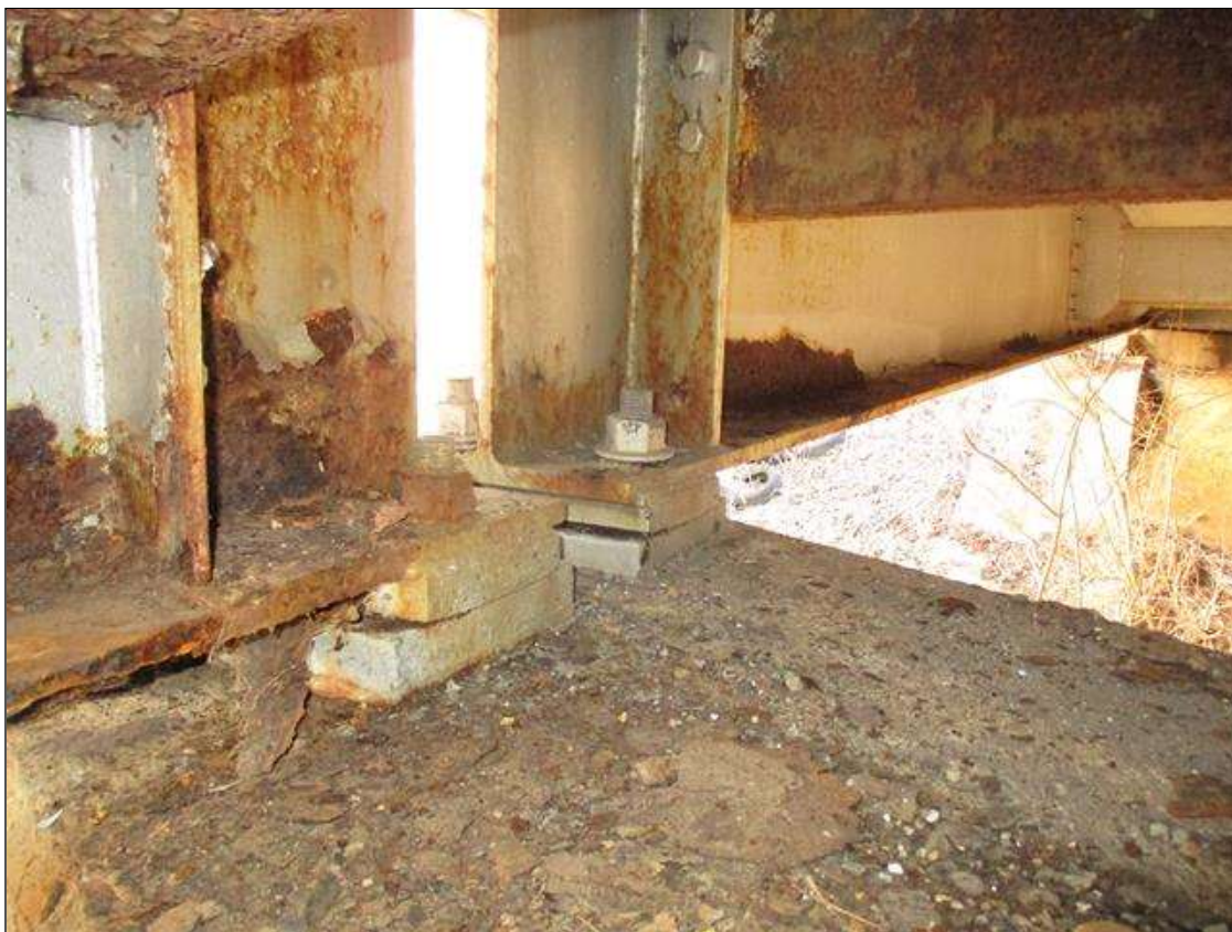
Span 3 Beam 1 - Near Bearing - Protective System: AREAS OF DETERIORATED PAINT SYSTEM THROUGHOUT BENT 1 BEARING
