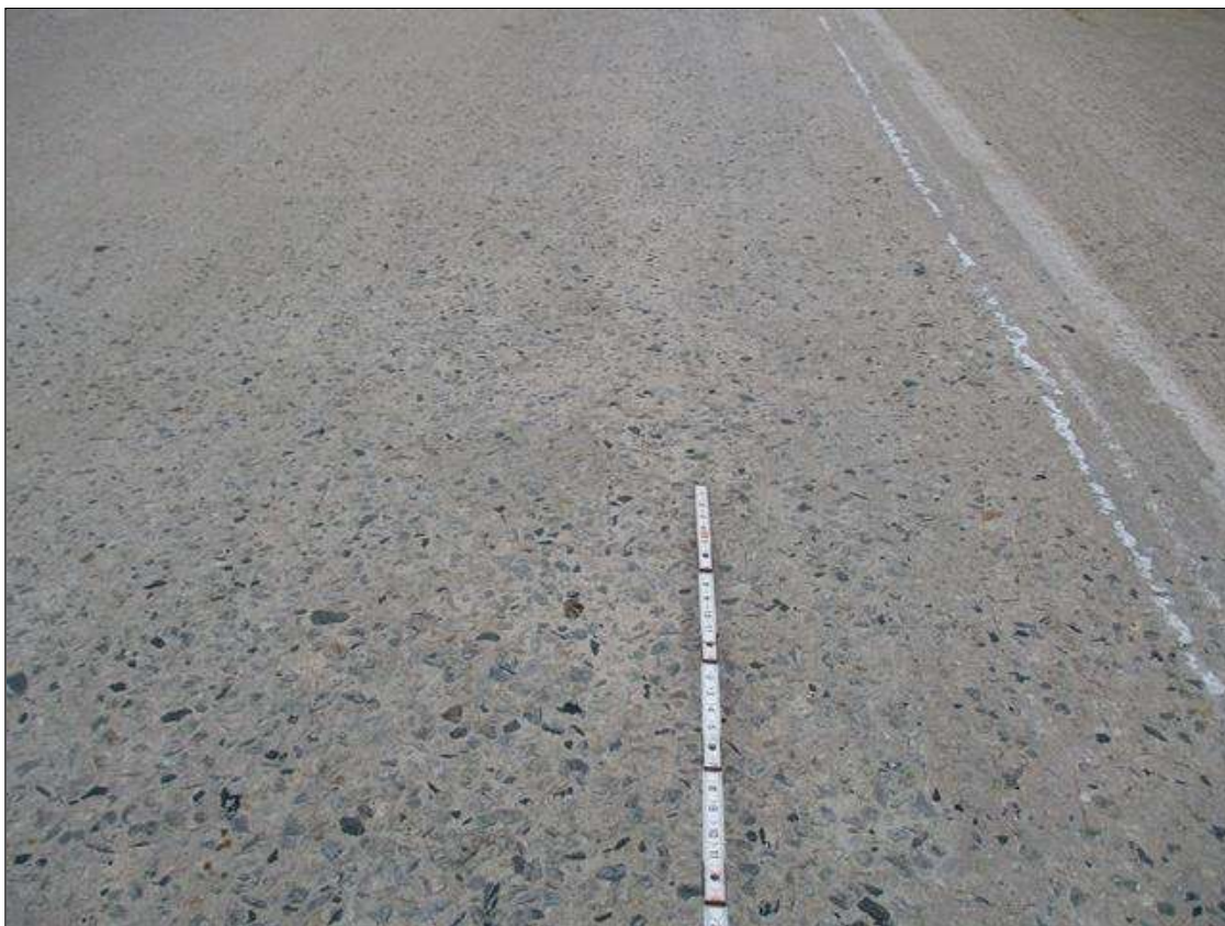
Span 3 Deck: SCALING WITH EXPOSED AGGREGATE IN TOP OF DECK THROUGHOUT TRAVEL LANES
