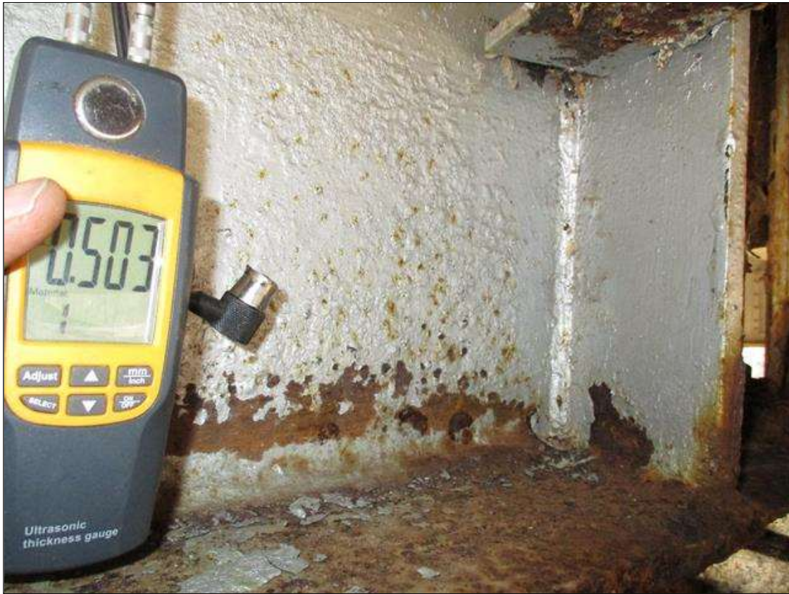
Span 3 Beam 3: (PAR) CORROSION ALONG BOTH FACES OF WEB AND BOTTOM FLANGE UP TO 15" LONG X 5" HIGH DOWN TO 0.503" RESIDUAL WEB, AND 18" LONG X 11 3/4" WIDE DOWN TO 0.199" RESIDUAL FLANGE AT BENT 3 BEARING
