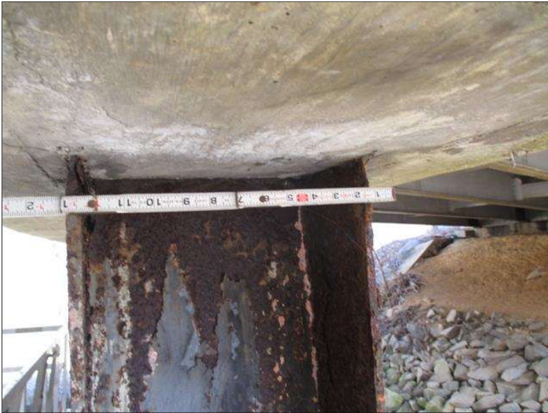
Bent 3 Pile 8: (PAR) CORROSION ALONG BOTH FLANGES UP TO 8" HIGH X 12" WIDE DOWN TO 1/8" RESIDUAL FLANGE AT BOTTOM OF CAP
