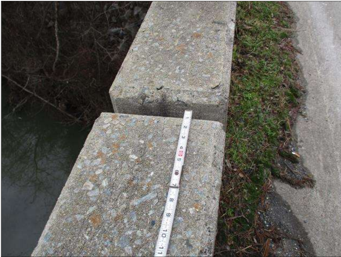
Span 2 Right Bridge Rail: UP TO 0.02" LONGITUDINAL CRACKS IN TOP OF RAIL IN VARIOUS LOCATIONS
