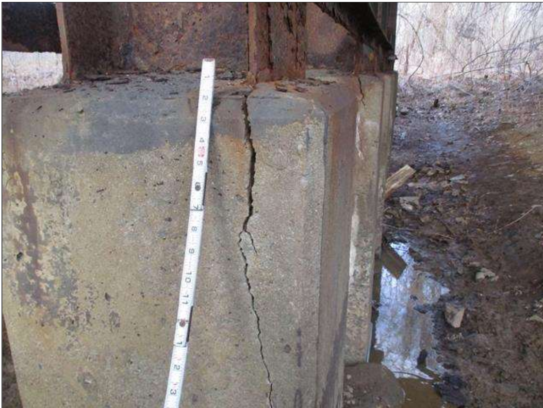
UP TO 3/8" TRANSVERSE AND VERTICAL CRACKS WITH AND WITHOUT EFFLORESCENCE IN ENCASEMENT (BENT 3, PILE 7)
