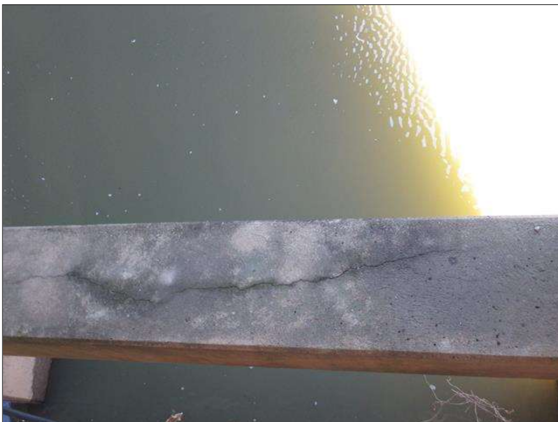
CRACKING IN TOP OF PILE BETWEEN 2 & 3 UP TO 1/4"
