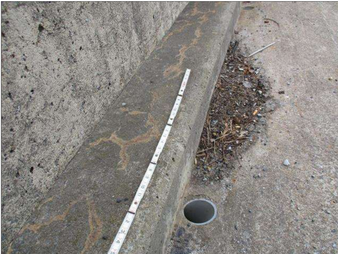
Span 1 Left Bridge Rail: ON TOP OF CURB THROUGHOUT, LESS THAN 0.01" WIDE CRACKING WITH EFFLORESCENCE
