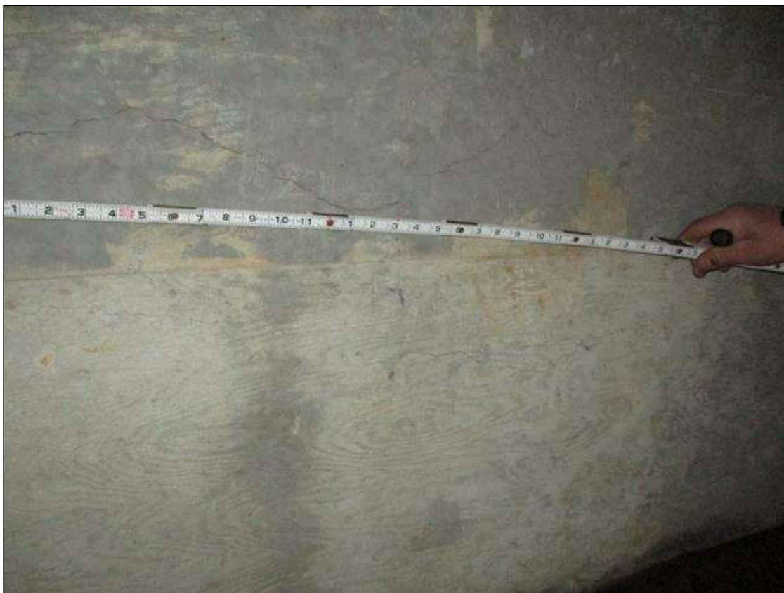
End Bent 2 Abutment: UP TO 0.02" HORIZONTAL AND MAP CRACKS THROUGHOUT FACE OF CURTAIN WALL IN BAYS 1 THRU 5
