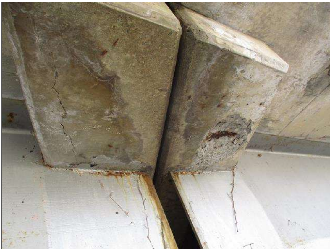
Span 3 Deck: 12"x 12"x 1" SPALL WITH EXPOSED REBAR BENT 3, LEFT SIDE, UNDERSIDE OF DECK
