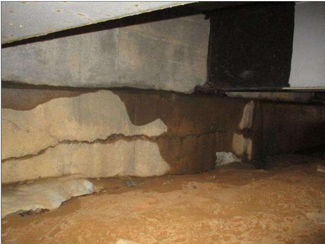
End Bent 2 Cap 1: UP TO 0.016" LONGITUDINAL AND HORIZONTAL CRACKS AND HAIRLINE MAP CRACKS WITH EFFLORESCENCE IN TOP AND FACE OF CAP AND BRACE PILE CAP AT LEFT END
