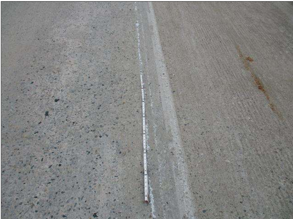
Span 3 Deck: 31" X 1/8" TRANSVERSE CRACK IN TOP OF DECK IN WESTBOUND LANE, APPROXIMATELY 14' FROM BENT 3 JOINT
