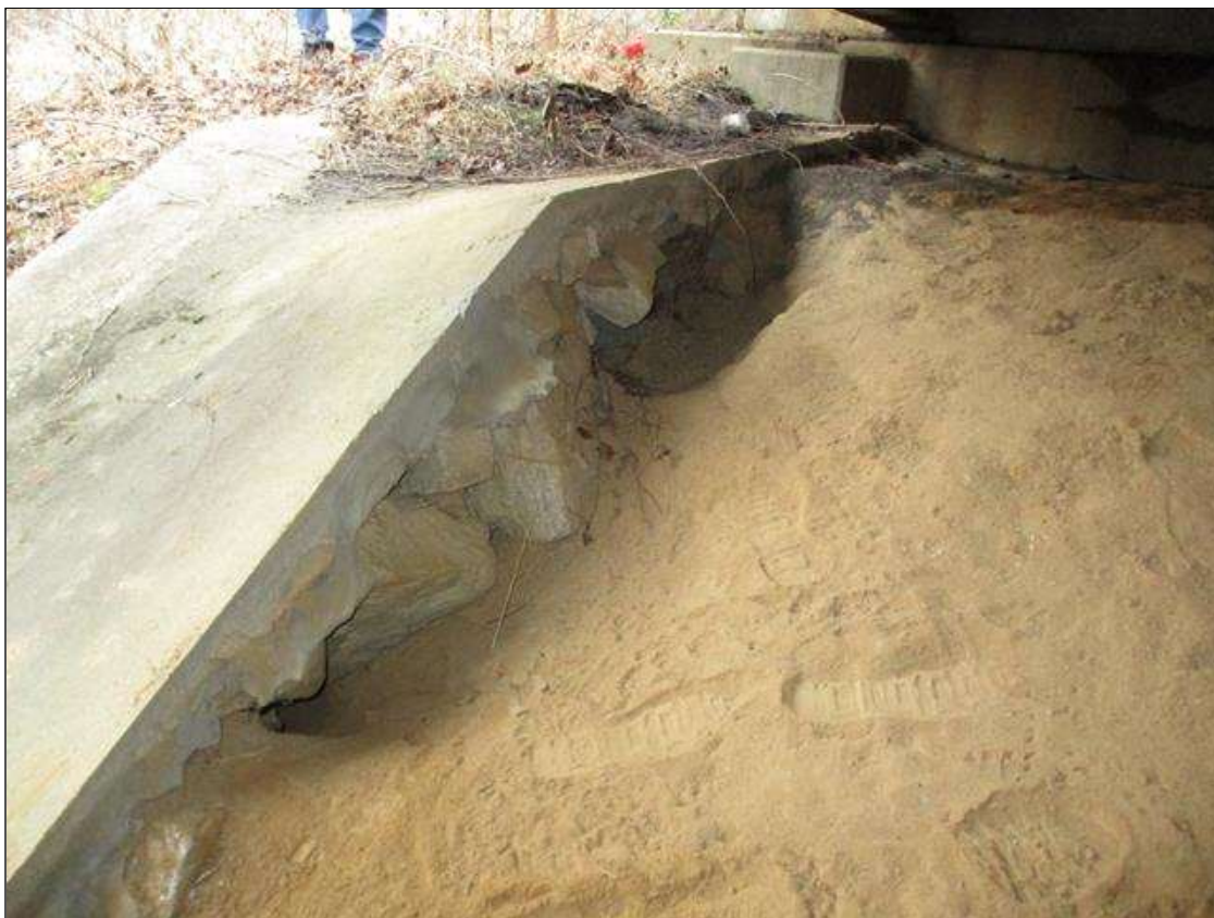
(PAR) END BENT 2 SLOPE PROTECTION, ALONG LEFT CONCRETE CHUTE; UP TO 3' DEEP X 8' LONG EROSION OF SOIL
