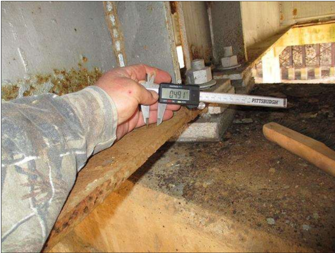
Span 1 Beam 4: (PAR) CORROSION ALONG RIGHT FACE OF WEB AND BOTTOM FLANGE UP TO 36" LONG X 4" HIGH WITH NO MEASURABLE LOSS OF SECTION BENEATH PAINT REPAIR IN WEB, AND 20" LONG X 5" WIDE DOWN TO .49" RESIDUAL FLANGE, APPROXIMATELY 4" FROM FACE OF BENT 1 BEARING
