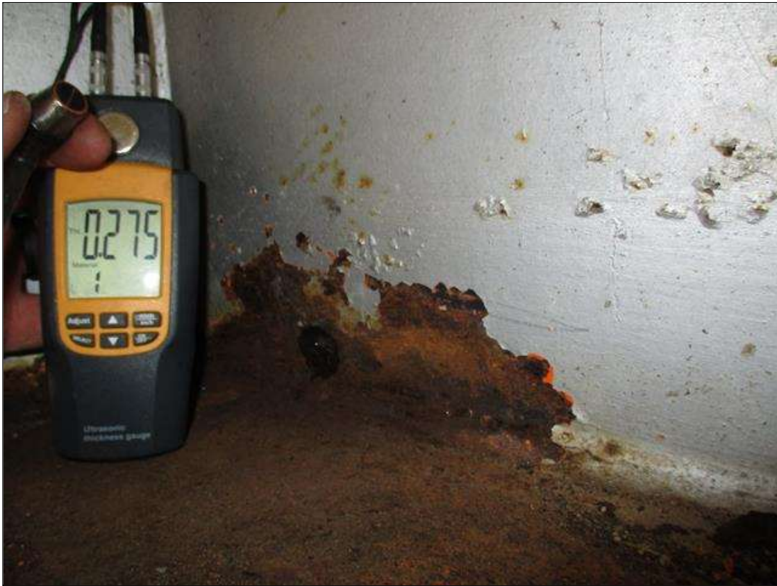
Span 2 Beam 2: (PAR) CORROSION ALONG BOTH FACES OF WEB AND BOTTOM FLANGE UP TO 33" LONG X 6" HIGH DOWN TO 0.275" RESIDUAL WEB, AND 34" LONG X 5" WIDE DOWN TO .328" RESIDUAL FLANGE AT BENT 2 BEARING
