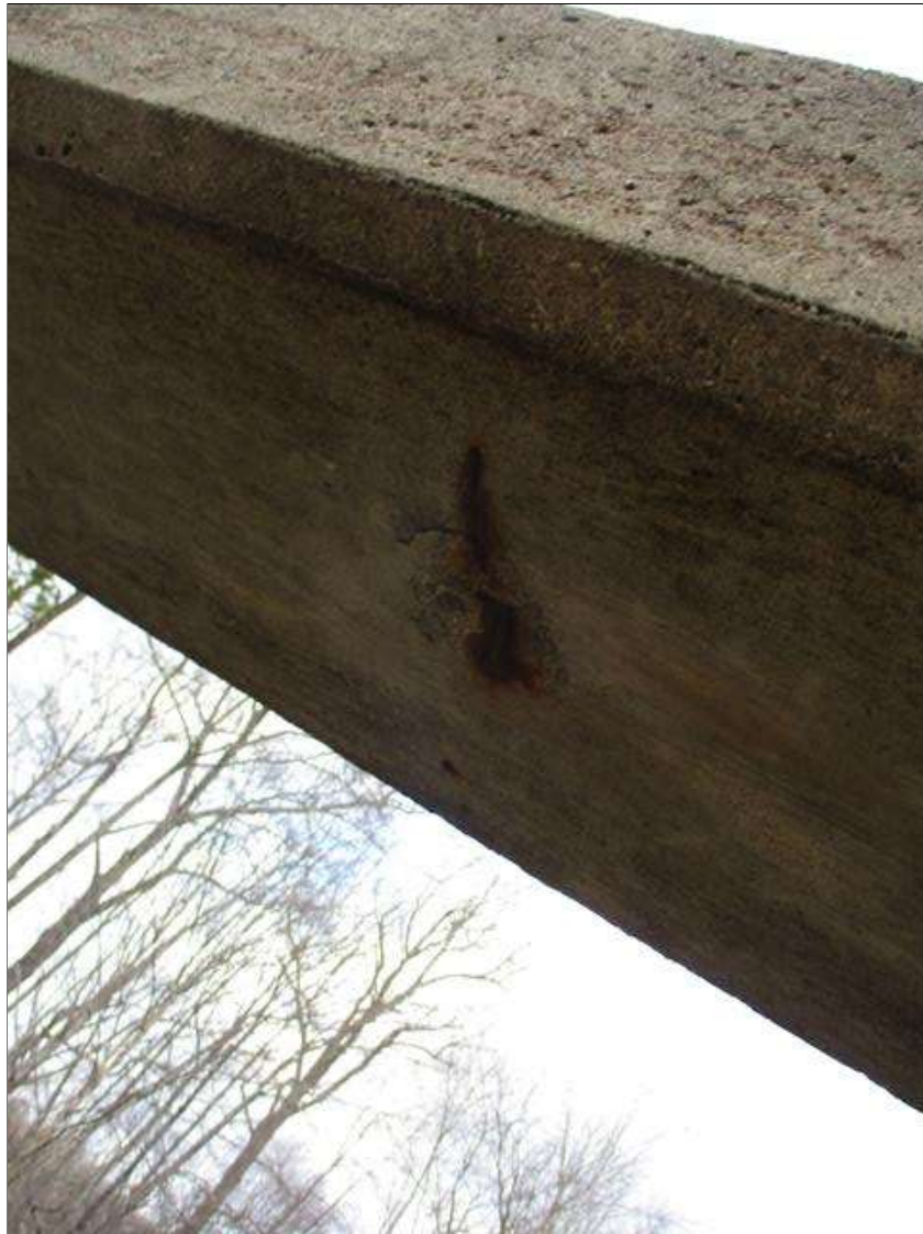
Span 2 Left Bridge Rail: THREE (3) SPALLS WITH EXPOSED REBAR UP TO 5" X 3" X 3/4" DEEP IN BOTTOM OF RAIL IN VARIOUS LOCATIONS
