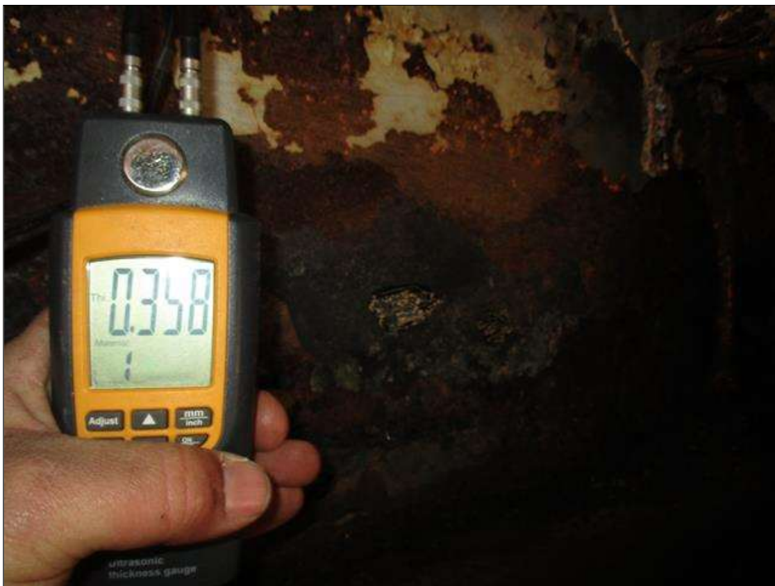
Span 4 Beam 5: (PAR) CORROSION ALONG BOTH FACES OF WEB AND BOTTOM FLANGE UP TO 105" LONG X 19" HIGH DOWN TO 0.358" RESIDUAL WEB, AND 72" LONG X 11 3/4" WIDE DOWN TO 0.459" RESIDUAL FLANGE AT BENT 3 BEARING
