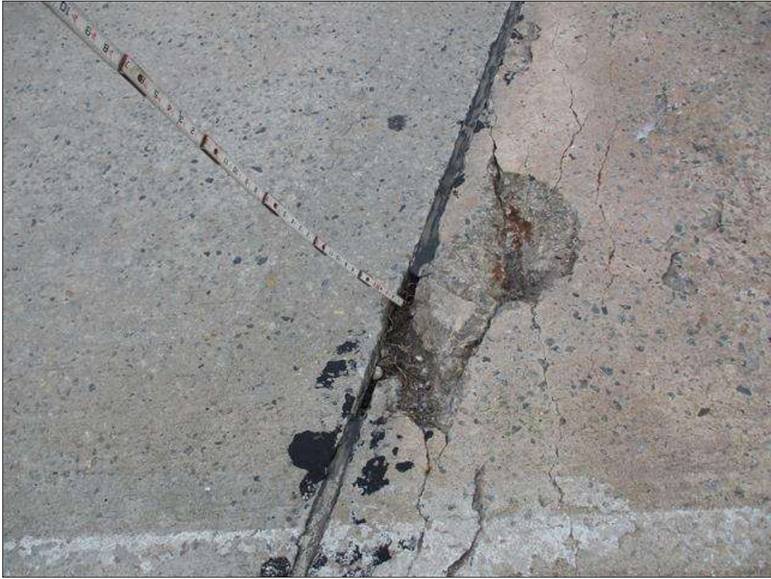
Span 4 Deck: (PAR) 15' X 11" X 3 1/2" DEEP SPALL WITH EXPOSED REBAR IN TOP OF DECK IN WHEEL LINE OF EASTBOUND LANE AT BENT 3 JOINT
