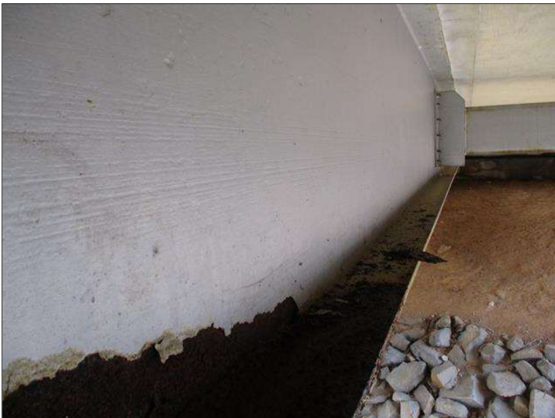
TYPICAL DETERIORATED PAINT SYSTEM (SPAN 4, BEAM 4)
