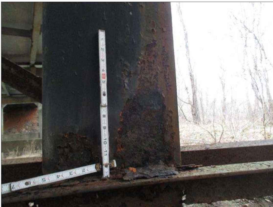
TYPICAL SURFACE CORROSION & DETERIORATED PAINT SYSTEM (BENT 3, PILE 3)
