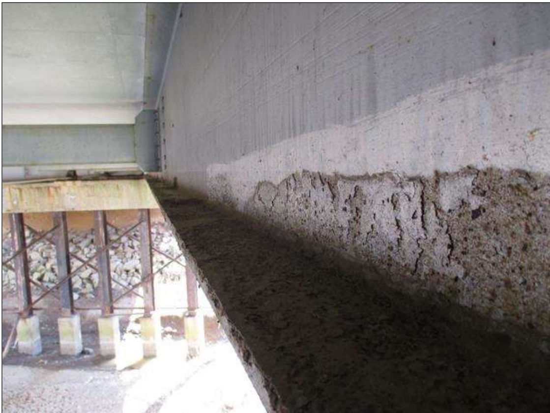
TYPICAL SURFACE CORROSION & DETERIORATED PAINT SYSTEM (SPAN 3, BEAM 5)
