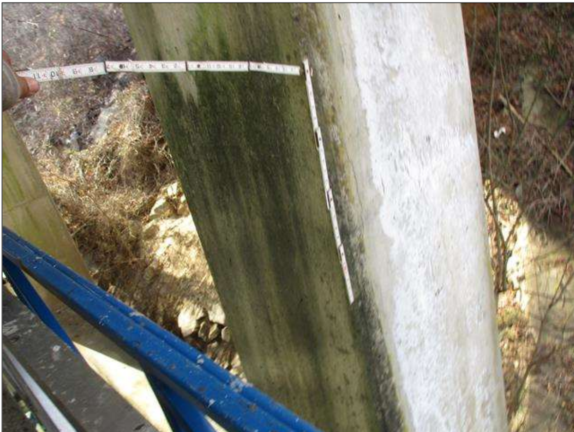
Bent 1 Pile 3: UP TO 8' X 0.03" VERTICAL CRACKS THROUGHOUT COLUMN
