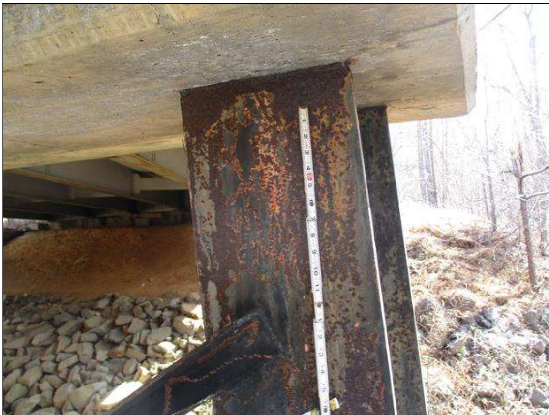
TYPICAL SURFACE CORROSION & DETERIORATED PAINT SYSTEM (BENT 3, PILE 10)
