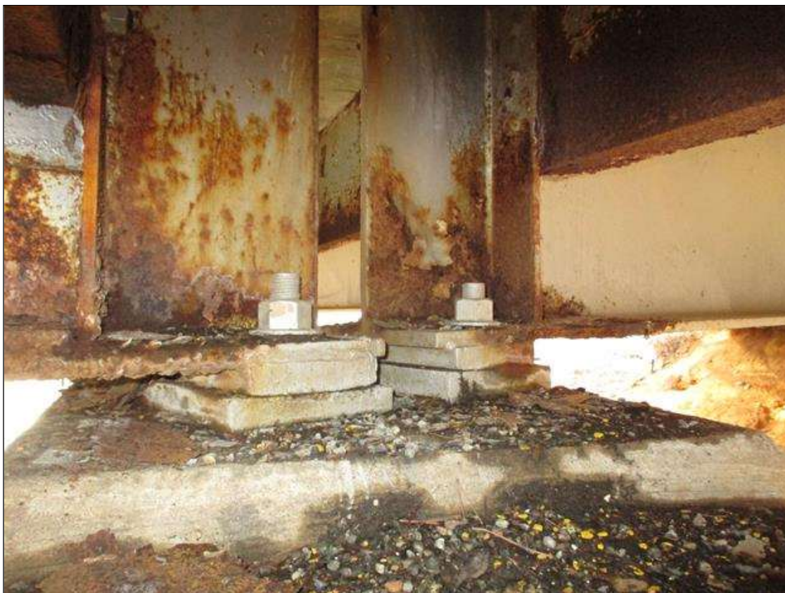
Span 1 Far Bearing: AREAS OF SURFACE CORROSION THROUGHOUT BEAM 1 BEARING
