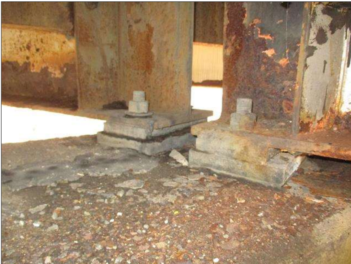
TYPICAL SURFACE CORROSION & DETERIORATED PAINT SYSTEM IN BEARINGS & BEAMS (SPAN 3, BEAMS 5 & 6)
