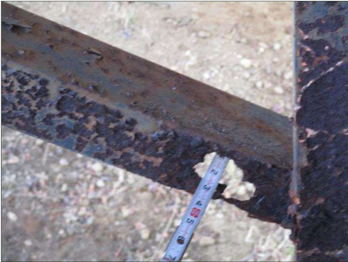
(PAR) AREAS OF 100% SECTION LOSS UP 17" X 3" AND BROKEN AND DETACHED CROSS BRACING INTERMITTENT THROUGHOUT BENT 3
