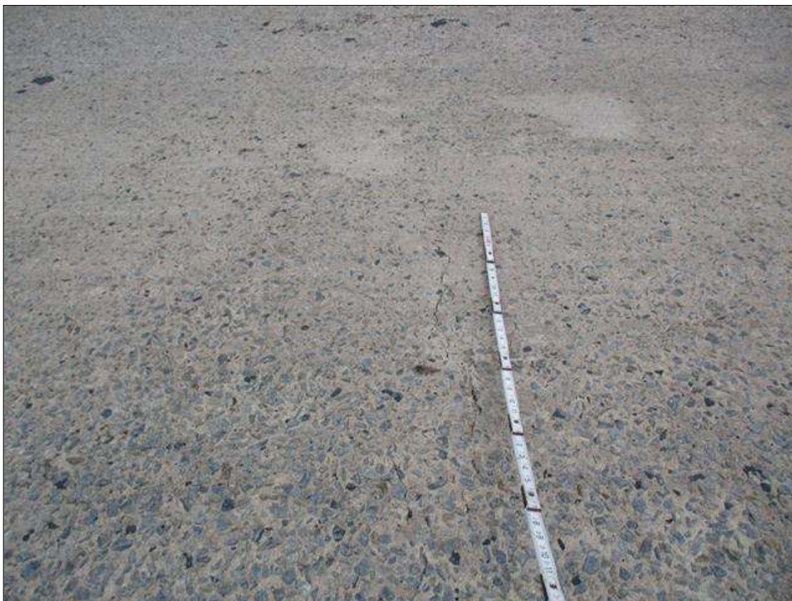
Span 4 Deck: UP TO 0.035" TRANSVERSE CRACKS IN TOP OF DECK IN TRAVEL LANES AT BENT 3 JOINT
