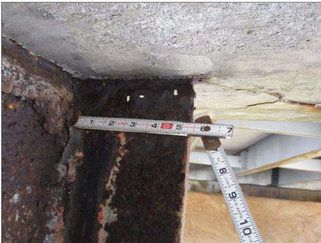
Bent 3 Pile 4: (PAR) CORROSION ALONG BOTH FLANGES UP TO 5" HIGH X 12" WIDE, 100% SECTION LOSS ON FLANGE AT BOTTOM OF CAP
