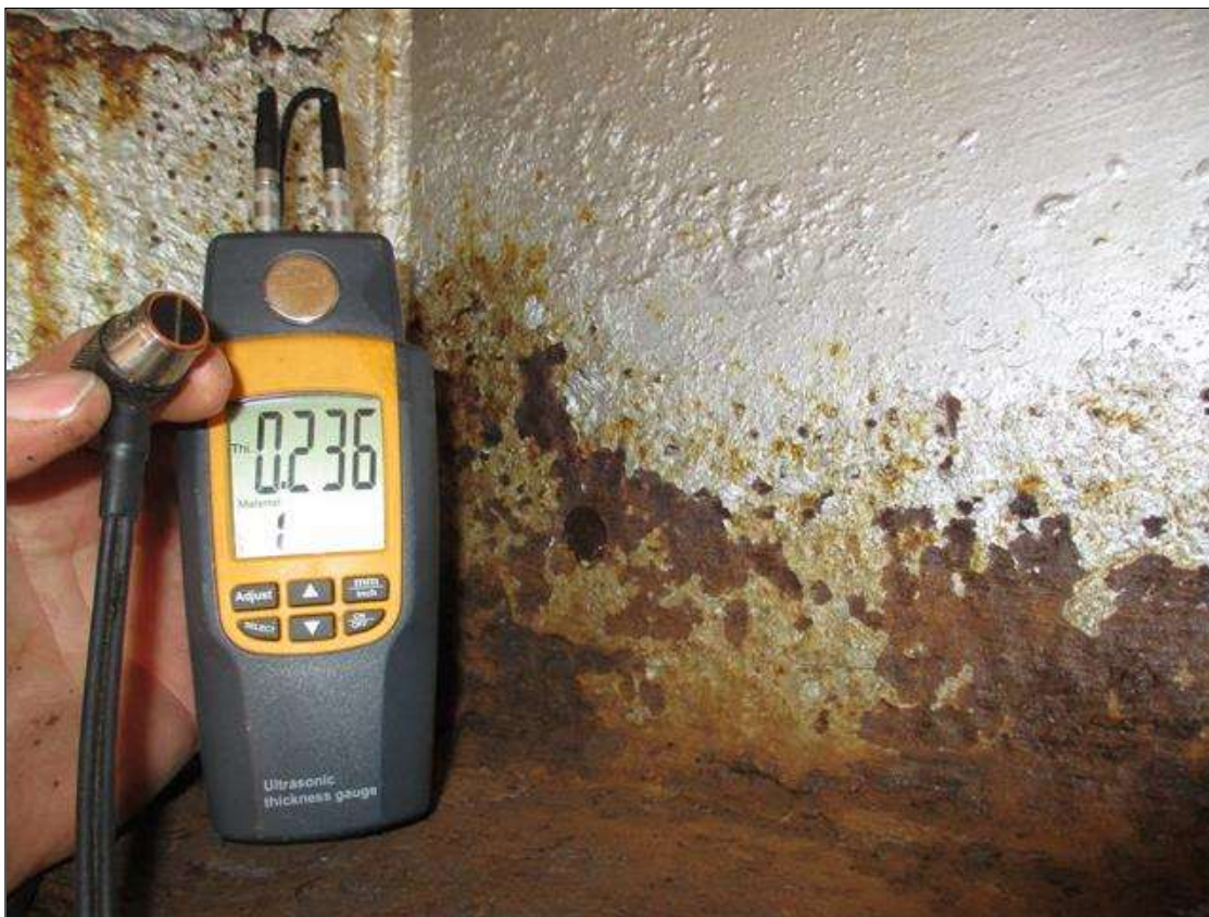
Span 4 Beam 3: (PAR) CORROSION ALONG BOTH FACES OF WEB AND BOTTOM FLANGE UP TO 14" LONG X 8" HIGH DOWN TO 0.236" RESIDUAL WEB, AND 24" LONG X 11 3/4" WIDE DOWN TO 0.200" RESIDUAL FLANGE AT BENT 3 BEARING
