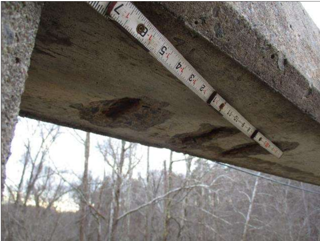
Span 4 Right Bridge Rail: THREE (3) SPALLS WITH EXPOSED REBAR UP TO 5" X 3 1/2" X 1/2" DEEP IN BOTTOM OF RAIL, APPROXIMATELY 14' FROM BENT 3 JOINT
