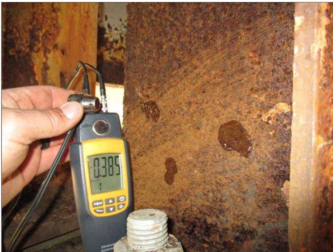
Span 3 Beam 3: (PAR) CORROSION ALONG LEFT FACE OF WEB AND BOTTOM FLANGE UP TO 72" LONG X 24" HIGH DOWN TO 0.385" RESIDUAL WEB, AND 72" LONG X 11 1/2" WIDE DOWN TO 0.360" RESIDUAL FLANGE AT BENT 2 BEARING (SEE PHOTOS)
