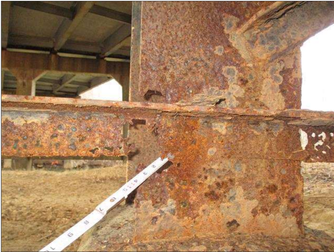
Bent 3 Pile 6: (PAR) CORROSION ALONG WEB AND BOTH FLANGES UP TO 19" HIGH X 11" WIDE WITH NO MEASURABLE LOSS OF SECTION IN WEB, AND 19" HIGH X 12" WIDE DOWN TO KNIFE'S EDGE RESIDUAL FLANGE WITH 2 LOCATIONS OF UP TO 6" HIGH X 3" WIDE 100% LOSS OF SECTION ABOVE CONCRETE ENCASEMENT
