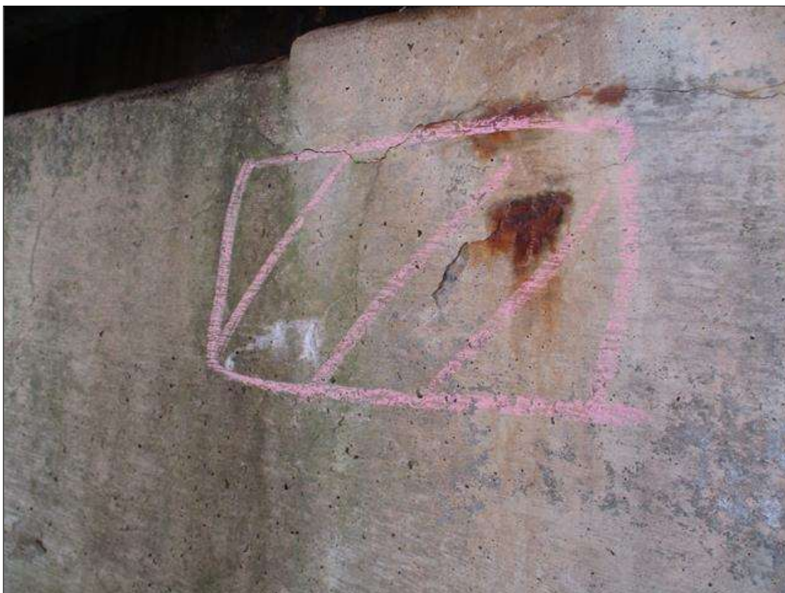
Bent 2 Cap 1: NEAR FACE, ABOVE COLUMN 2, DELAMINATED AREA 2' HIGH X 8" WIDE
