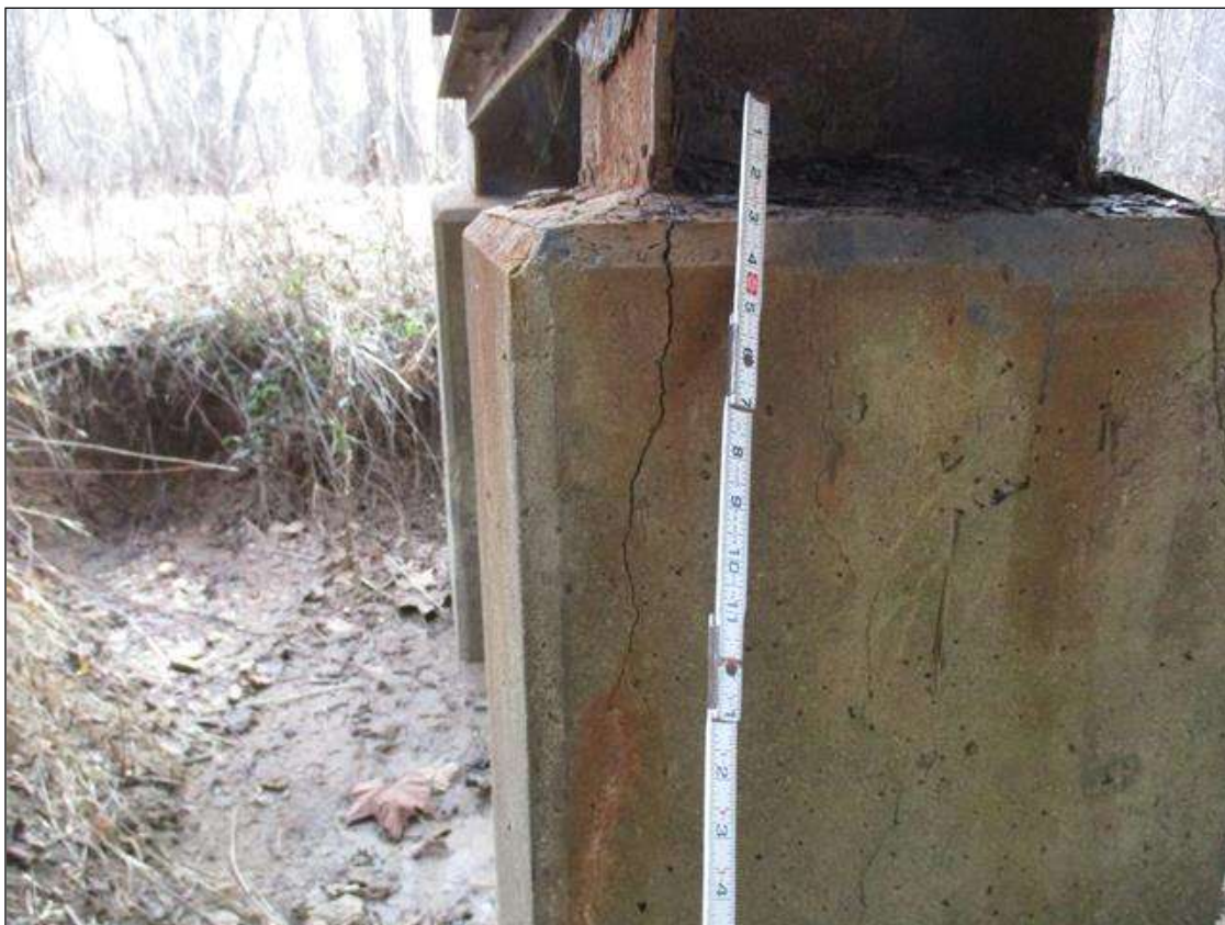
UP TO 1/8" TRANSVERSE & VERTICAL CRACKS WITH AND WITHOUT EFFLORESCENCE IN ENCASEMENT
