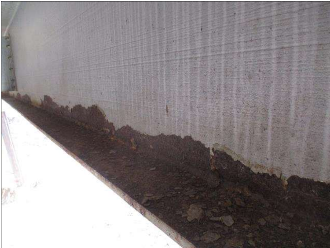
TYPICAL DETERIORATED PAINT SYSTEM (SPAN 3, BEAM 6)
