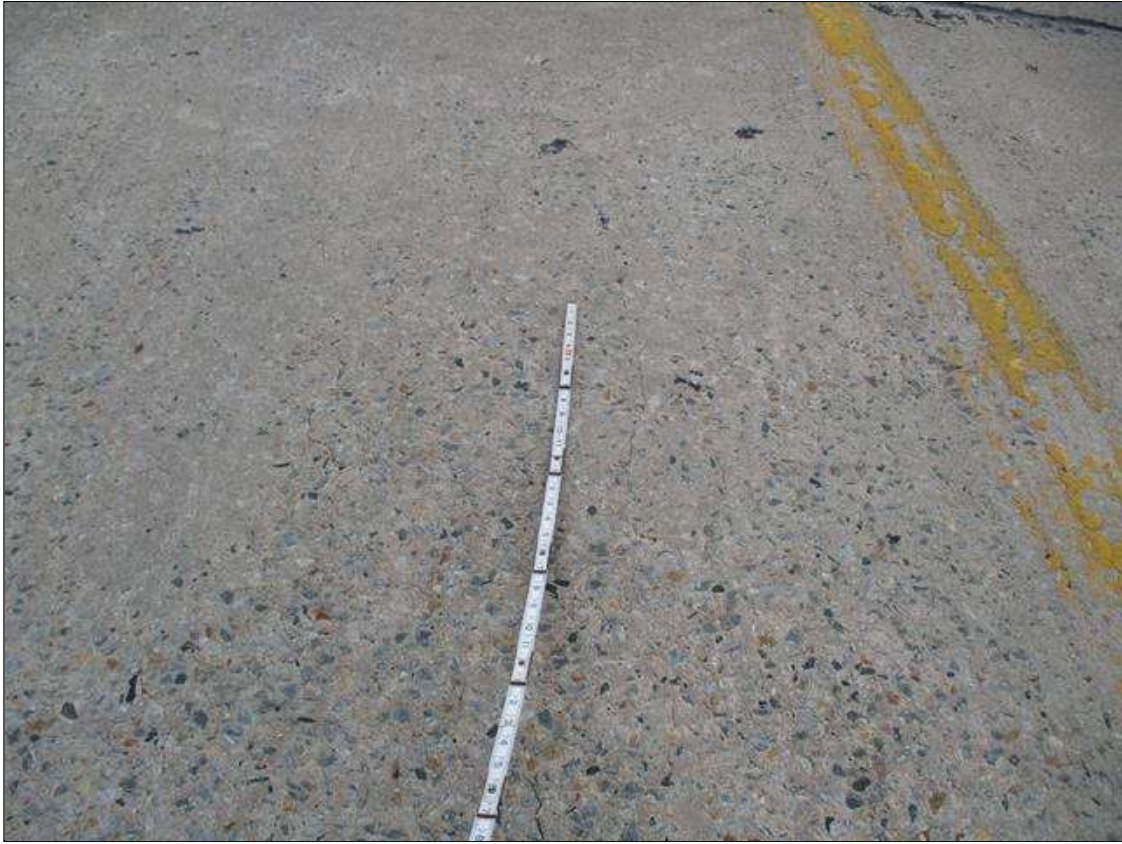
Span 1 Deck: UP TO 0.02" MAP CRACKS THROUGHOUT TOP OF DECK
