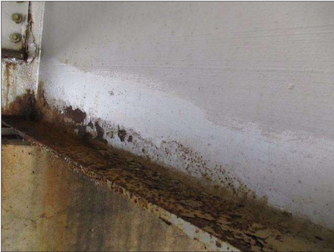
TYPICAL SURFACE CORROSION & DETERIORATED PAINT SYSTEM (SPAN 4, BEAM 3)
