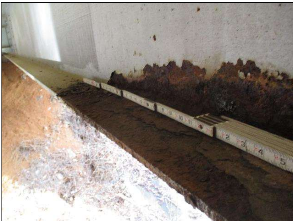
TYPICAL DETERIORATED PAINT SYSTEM SPAN 1, BEAM 2
