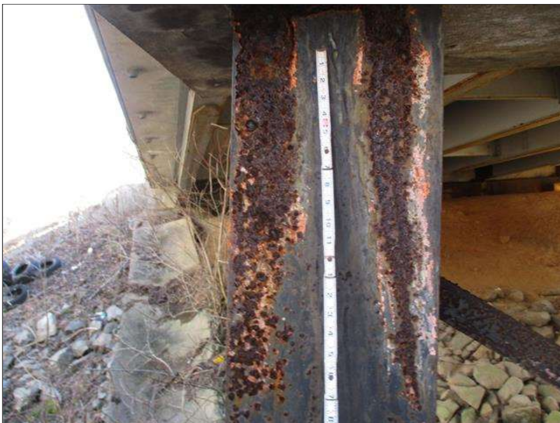
TYPICAL DETERIORATED PAINT SYSTEM (BENT 3, PILE 1)
