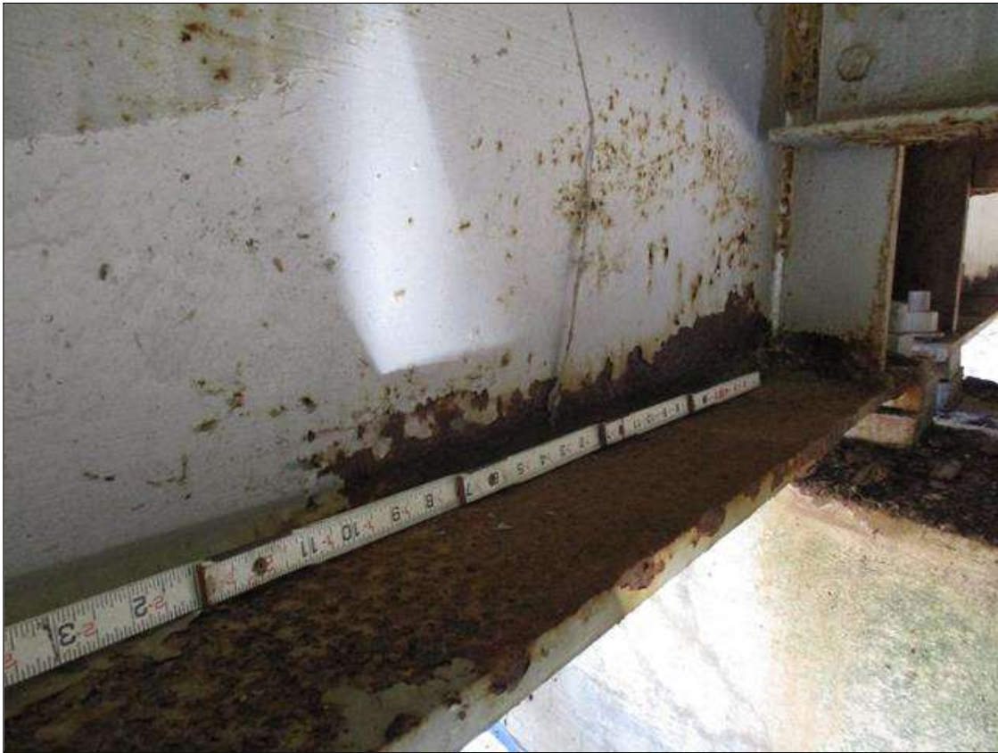
TYPICAL CORROSION (SPAN 2, BEAM 1)
