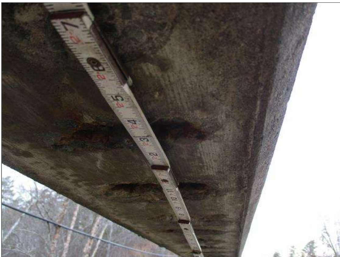
Span 3 Right Bridge Rail: SPALLS WITH EXPOSED REBAR UP TO 6" X 4" X 1/4" DEEP IN BOTTOM OF RAIL IN VARIOUS LOCATIONS
