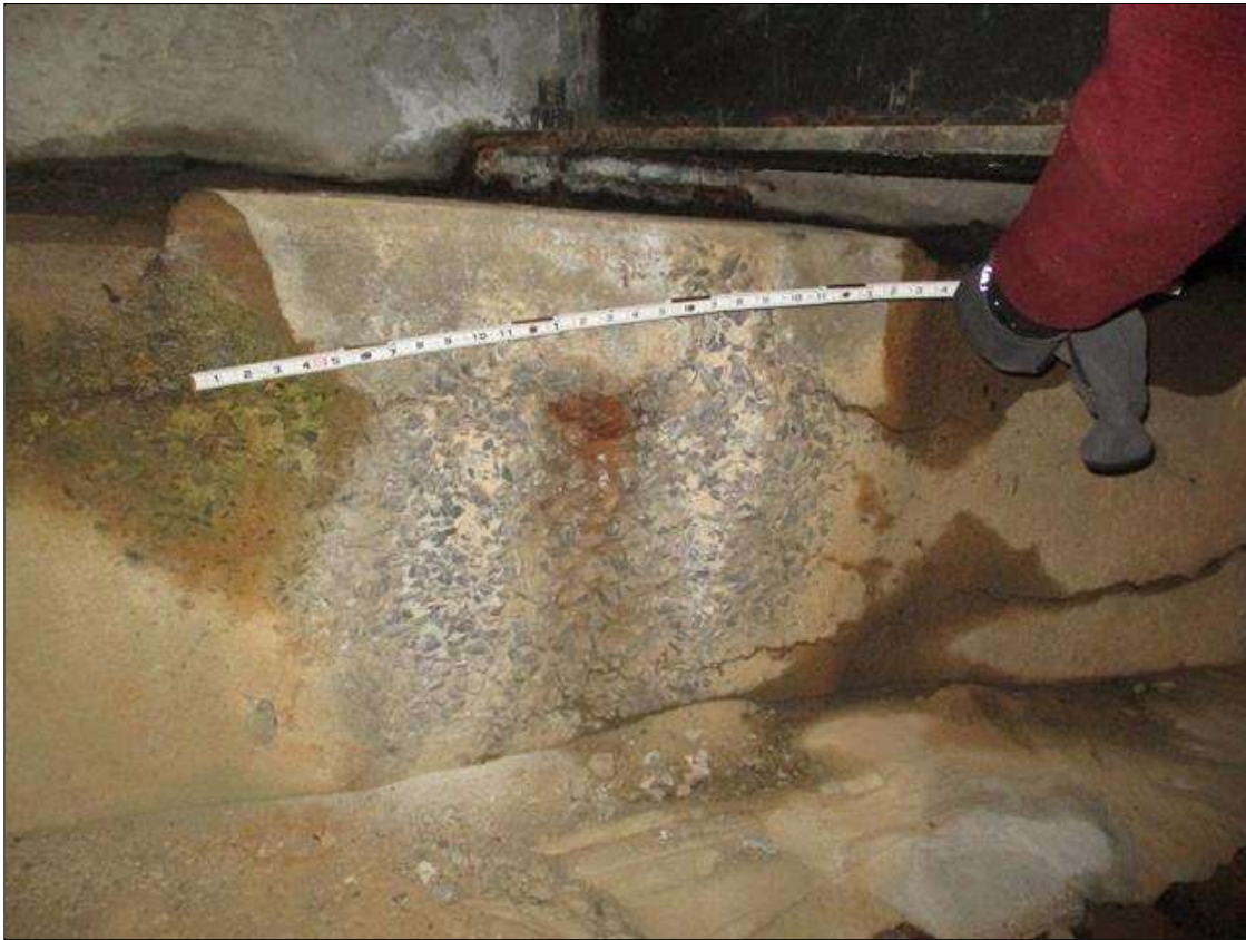
End Bent 2 Cap 1: 105" X 23" SECTION OF UP TO 22" X 20" AREAS OF SCALING WITH EXPOSED AGGREGATE IN FACE OF CAP AND BRACE PILE CAP BENEATH BAY 3
