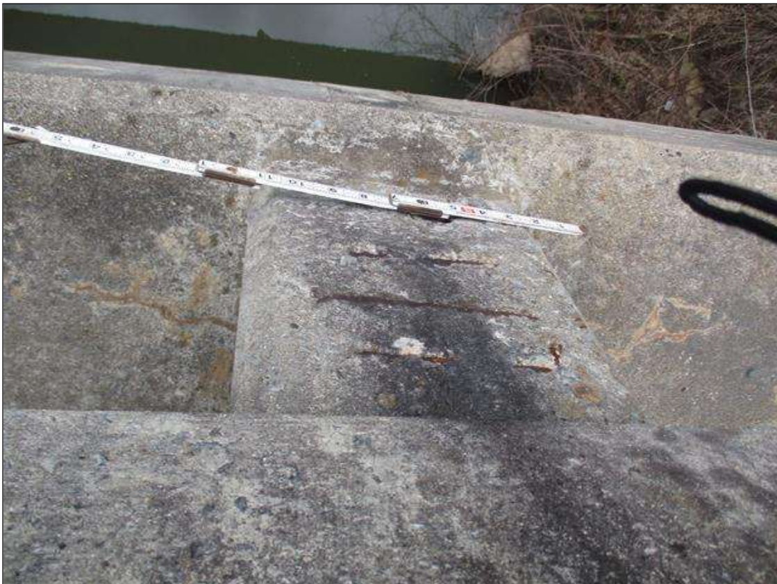
Span 2 Right Bridge Rail: SPALLS WITH EXPOSED REBAR UP TO 5" X 3" X 1/2" DEEP IN BOTTOM OF RAIL AND OUTSIDE FACES OF POSTS INTERMITTENT THROUGHOUT
