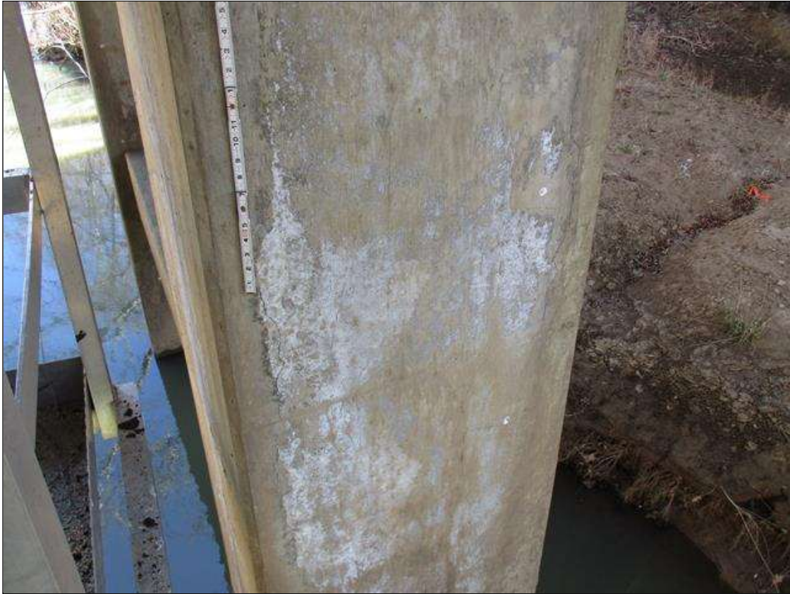
Bent 2 Pile 2: UP TO 18' X 1/16" VERTICAL CRACKS THROUGHOUT COLUMN, CRACK IN SPAN 2 FACE SHOWN IN PHOTO
