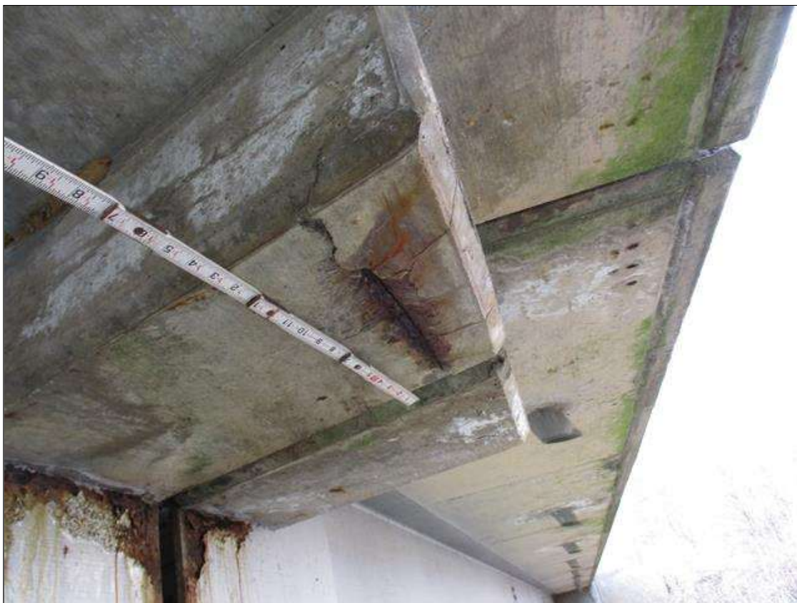
CONCRETE DIAPHRAGM, LEFT SIDE OF SPAN 2 BEAM 1 AT BENT 1, 12" LONG X 0.75" DEEP SPALL WITH EXPOSED REBAR WITH ACTIVE SECTION LOSS
