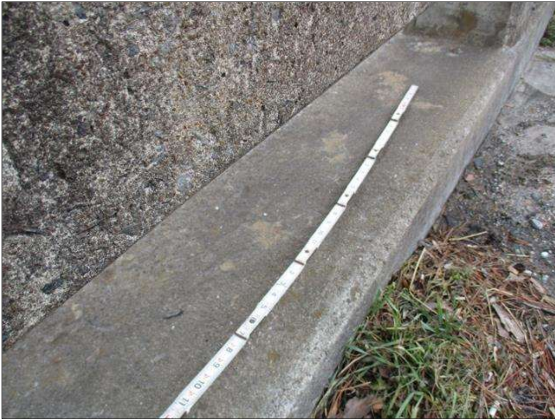
Span 3 Right Bridge Rail: ON TOP OF CURB THROUGHOUT, LESS THAN 0.01" WIDE CRACKING WITH EFFLORESCENCE
