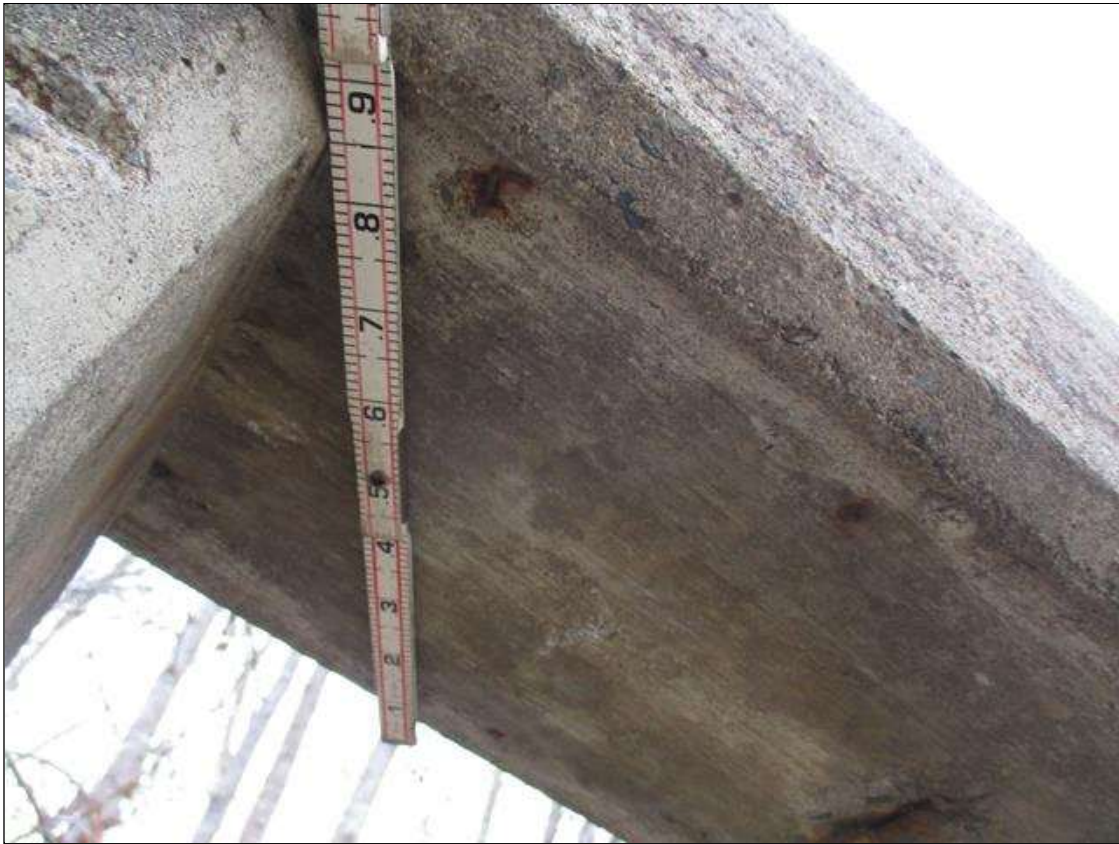
Span 4 Left Bridge Rail: FIVE (5) SPALLS WITH EXPOSED REBAR UP TO 5" X 4" X 1/2" DEEP IN BOTTOM OF RAIL IN VARIOUS LOCATIONS
