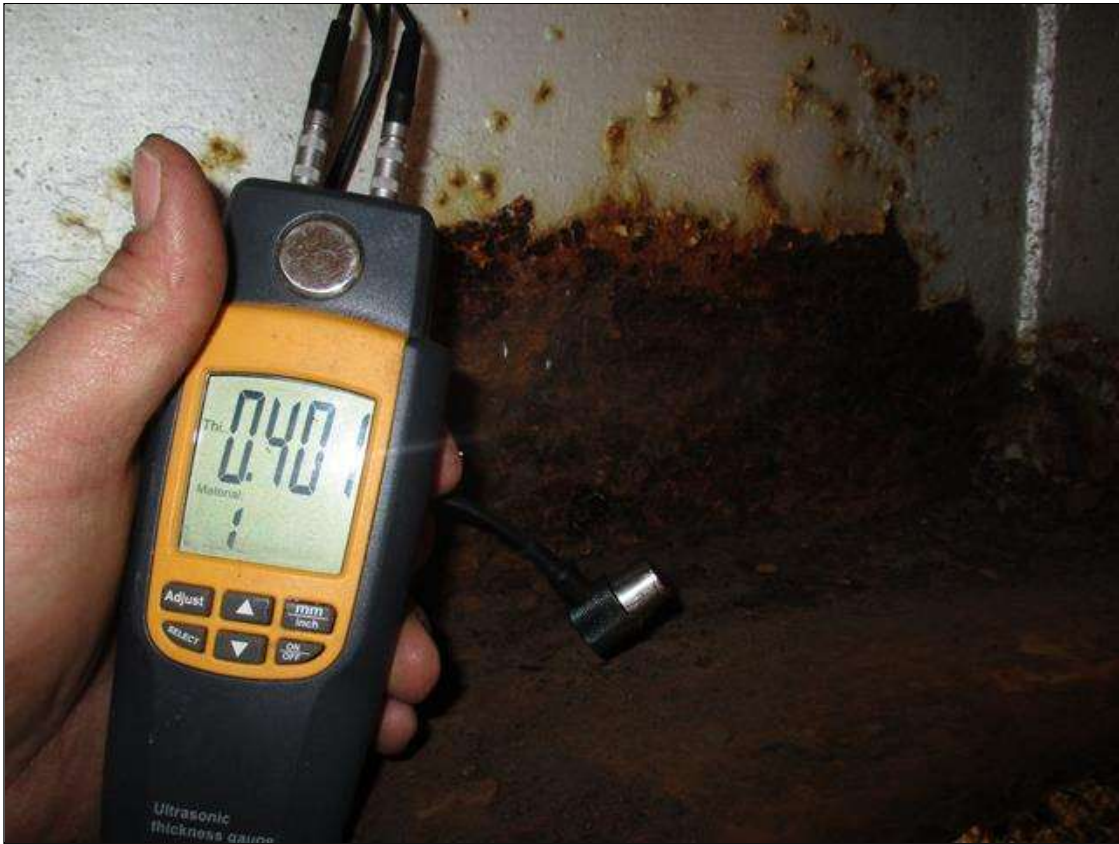
Span 3 Beam 1: (PAR) CORROSION ALONG RIGHT FACE OF WEB AND BOTTOM FLANGE UP TO 34" LONG X 5" HIGH DOWN TO 0.470" RESIDUAL WEB, AND 36" LONG X 5" WIDE DOWN TO 0.401" RESIDUAL FLANGE AT BENT 3 BEARING
