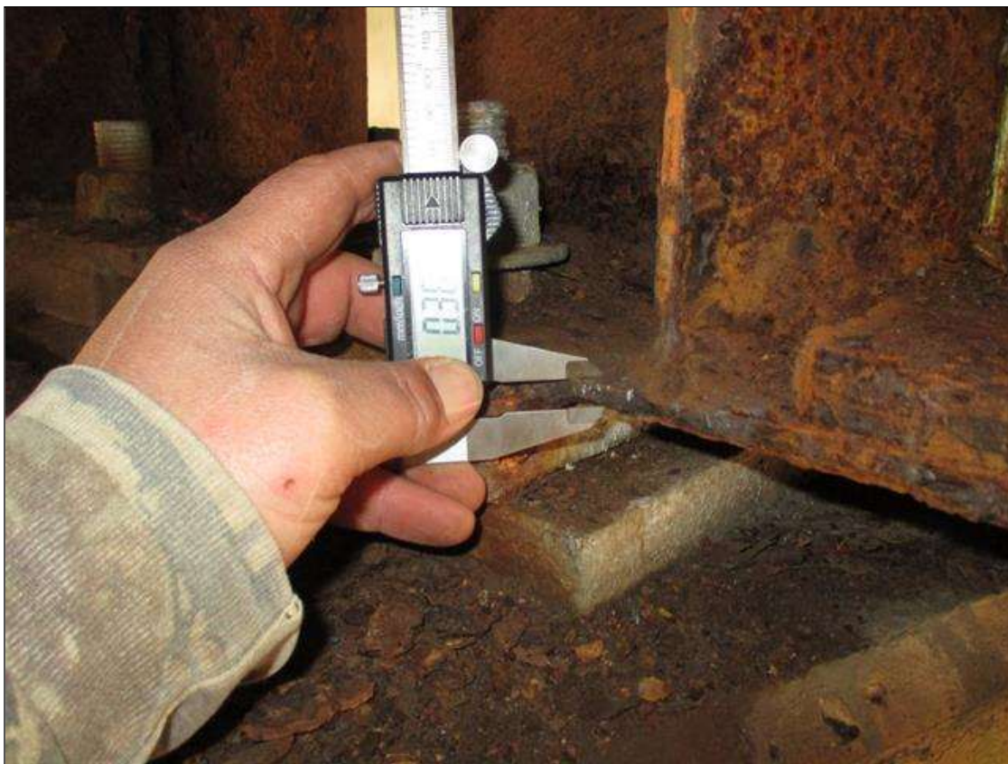
Span 3 Beam 3: (PAR) CORROSION ALONG LEFT FACE OF WEB AND BOTTOM FLANGE UP TO 72" LONG X 24" HIGH DOWN TO 0.385" RESIDUAL WEB, AND 72" LONG X 11 1/2" WIDE DOWN TO 0.360" RESIDUAL FLANGE AT BENT 2 BEARING (SEE PHOTOS)
