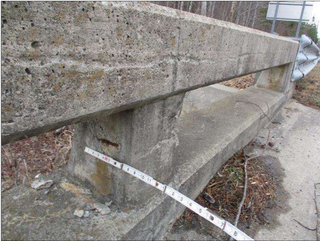
Span 1 Right Bridge Rail: 11" X 5" X 1/2" DEEP SPALL IN FACE OF RAIL, APPROXIMATELY 19' FROM END BENT 1 FILL FACE
