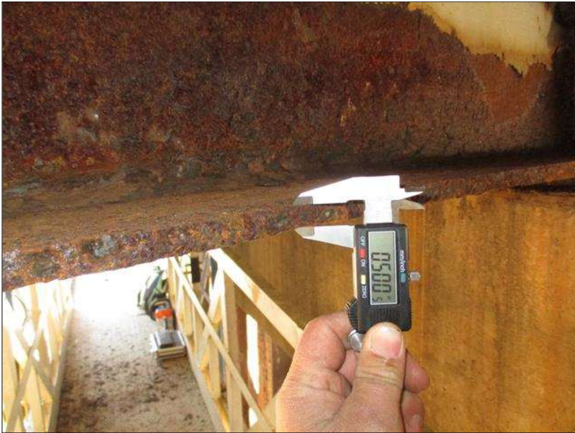
Span 4 Beam 4: (PAR) CORROSION ALONG BOTH FACES OF WEB AND BOTTOM FLANGE UP TO 108" LONG X 20" HIGH DOWN TO 0.393" RESIDUAL WEB, AND 103" LONG X 11 3/4" WIDE DOWN TO 0.500" RESIDUAL FLANGE AT BENT 3 BEARING
