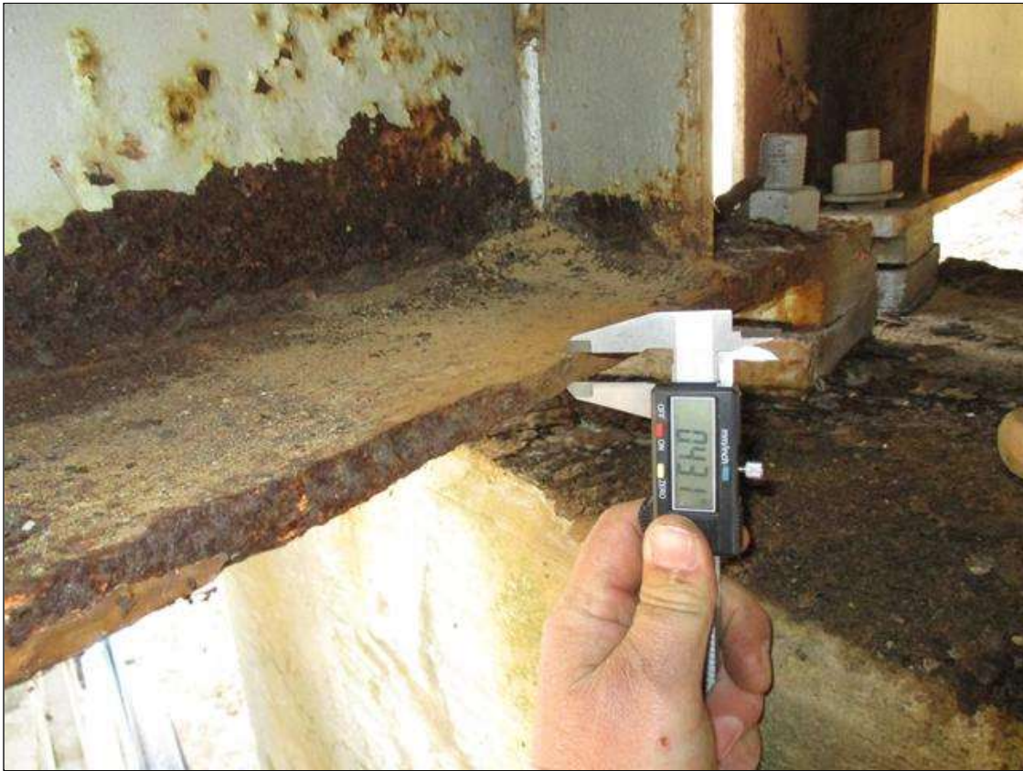
Span 2 Beam 1: (PAR) CORROSION ALONG BOTH FACES OF WEB AND BOTTOM FLANGE UP TO 36" LONG X 24" HIGH SURFACE CORROSION ON WEB, AND 36" LONG X 11 3/4" WIDE DOWN TO .431" RESIDUAL FLANGE AT BENT 2 BEARING
