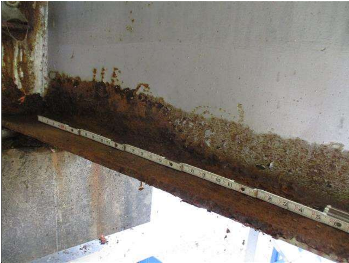
Span 2 Beam 1 - Protective System: DETERIORATED PAINT SYSTEM ALONG BOTH FACES OF WEB AND BOTTOM FLANGE UP TO 68" LONG X 10" HIGH IN WEB, AND 61" LONG X 11 3/4" WIDE IN FLANGE AT BENT 1 BEARING
