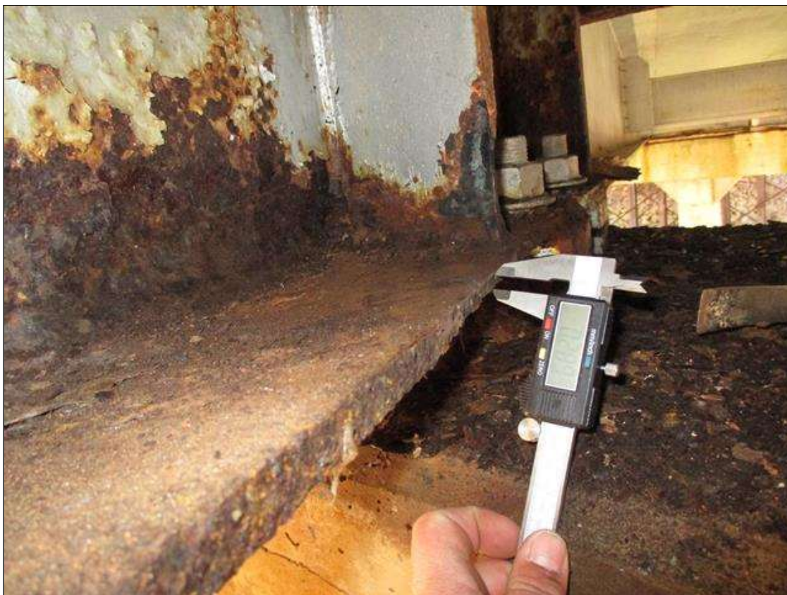
Span 1 Beam 3: (PAR) CORROSION ALONG BOTH FACES OF WEB AND BOTTOM FLANGE UP TO 34" LONG X 24" HIGH DOWN TO 0.291" RESIDUAL WEB, AND 36" LONG X 5" WIDE DOWN TO 0.289" RESIDUAL FLANGE AT BENT 1 BEARING
