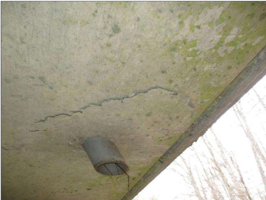
Span 1 Deck: UNDERSIDE, 17" X 12" AREA OF DELAMINATION IN BOTTOM OF LEFT OVERHANG AROUND DECK DRAIN AT BENT 1
