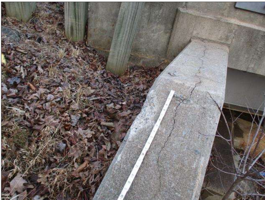
NEAR RIGHT WING, 3' LONGITUDINAL CRACK 0.0625" WIDE AND 6" X 3" X 0.5" DEEP SPALL ALONG TOP OF WALL
