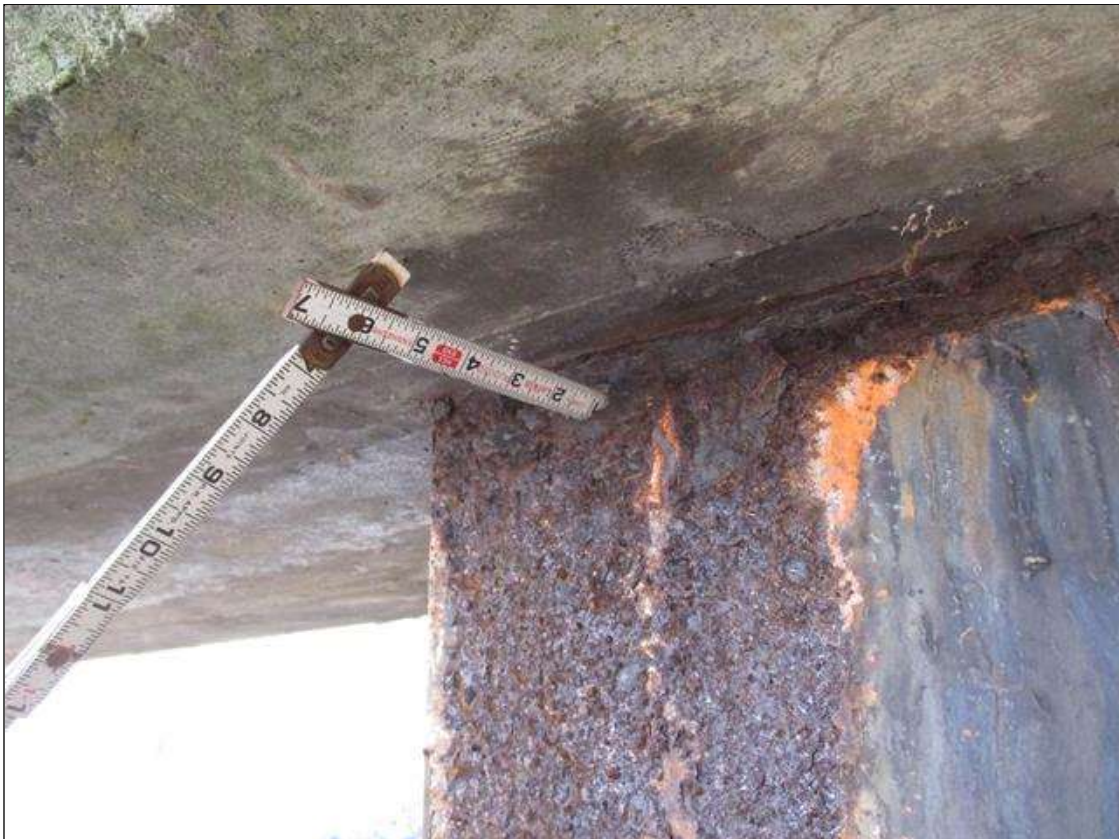
Bent 3 Pile 2: (PAR) CORROSION ALONG NEAR FLANGE UP TO 3" HIGH X 12" WIDE DOWN TO 1/4" RESIDUAL FLANGE WITH 3/16" DIAMETER HOLE AT BOTTOM OF CAP UP TO 3" LONG
