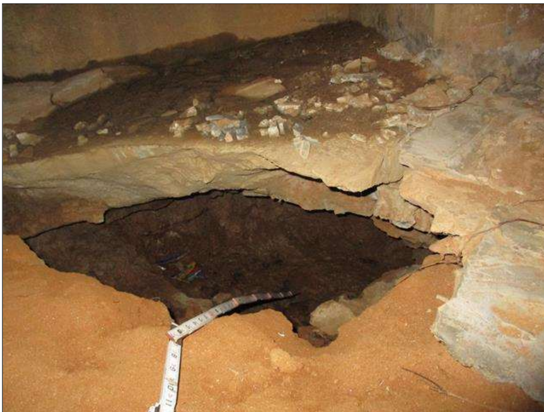
(PAR) SLOPE @ END BENT HAS EROSION AREA 5'x 8'x 4' DEEP UNDERMINING CAP BETWEEN BEAMS 1 & 2
