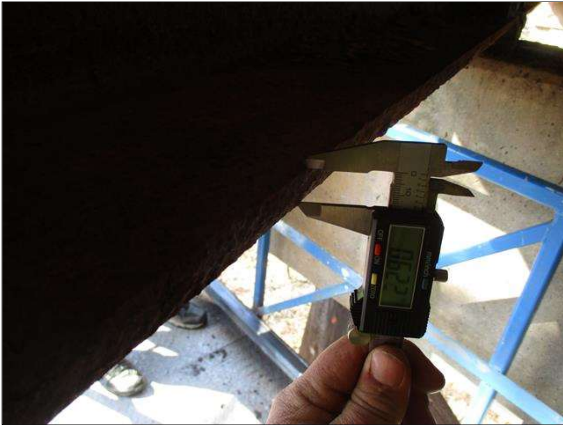
Span 4 Beam 6: CORROSION ON BOTTOM FLANGE, FULL WIDTH EXTENDING 5' FROM BENT 3, DOWN TO 0622" REMAINING FLANGE DEPTH
