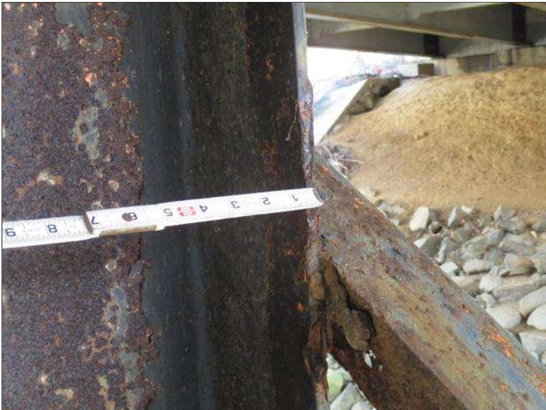
Bent 3 Pile 7: (PAR) CORROSION ALONG RIGHT EDGE OF FAR FLANGE UP TO 10" HIGH X 9" WIDE DOWN TO 1/4" RESIDUAL FLANGE, APPROXIMATELY 2' FROM BOTTOM OF CAP
