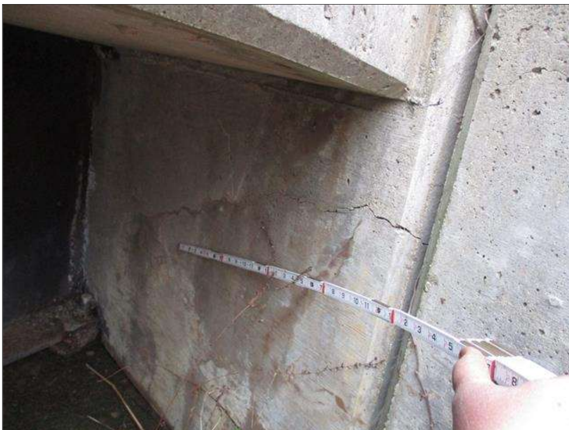
HORIZONTAL CRACKS AND HAIRLINE MAP CRACKS WITH EFFLORESCENCE IN FACE OF CURTAIN WALL (TYPICAL END BENT 2 ABUTMENT)
