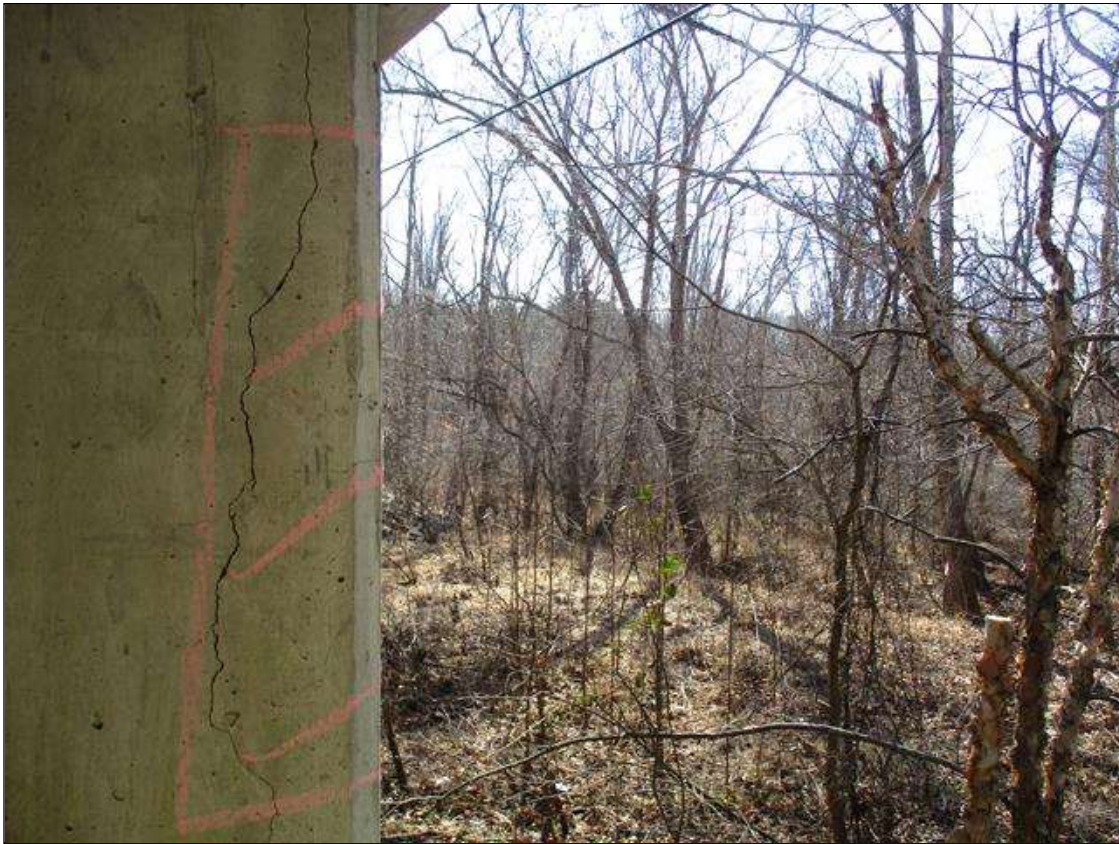
Bent 2 Pile 3: 22" X 5" X 5" AREA OF DELAMINATION WITH UP TO 0.05" VERTICAL CRACKS IN SOUTHWEST CORNER OF COLUMN, APPROXIMATELY 3' FROM BOTTOM OF CAP
