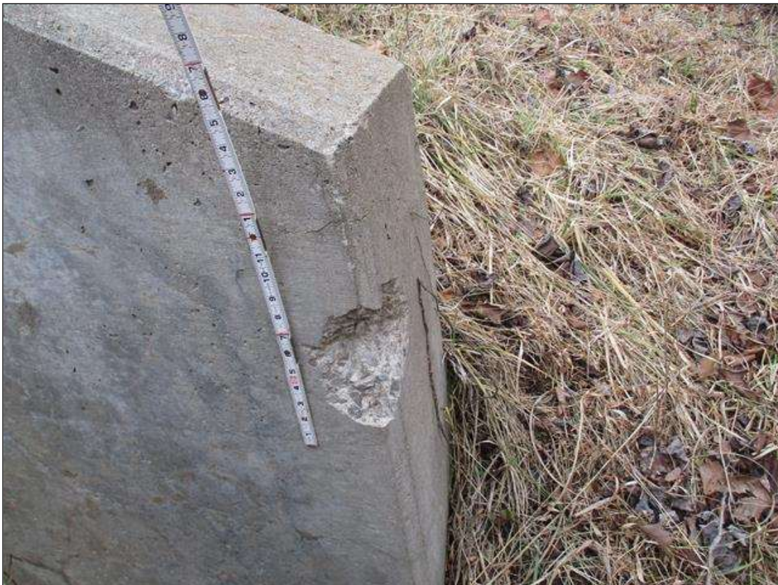
FAR RIGHT WING, 6" DIAMETER X 2" DEEP EDGE SPALL
