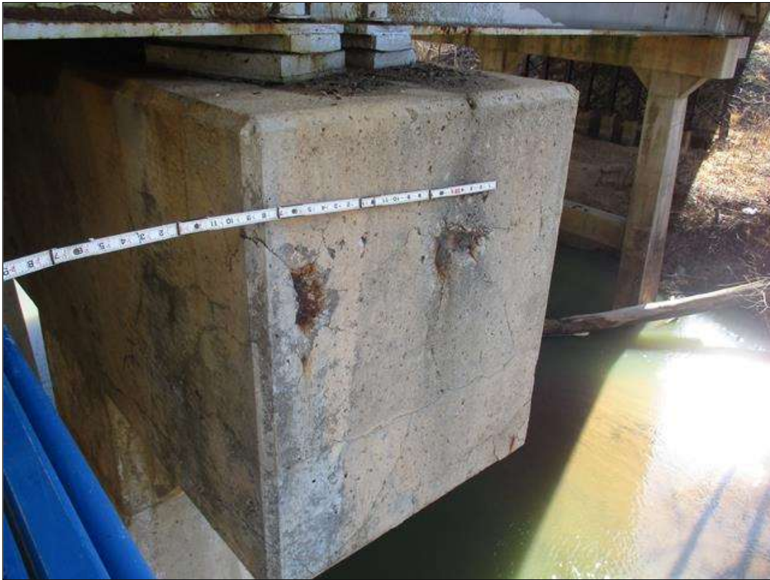
TYPICAL LONGITUDINAL, HORIZONTAL, MAP CRACKING & EXPOSED REBAR (BENT 1, CAP 1)
