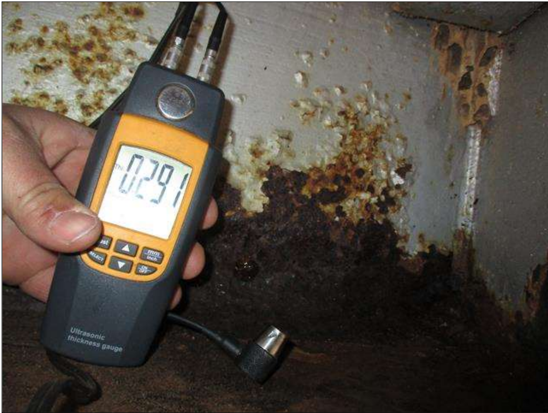
Span 1 Beam 3: (PAR) CORROSION ALONG BOTH FACES OF WEB AND BOTTOM FLANGE UP TO 34" LONG X 24" HIGH DOWN TO 0.291" RESIDUAL WEB, AND 36" LONG X 5" WIDE DOWN TO 0.289" RESIDUAL FLANGE AT BENT 1 BEARING
