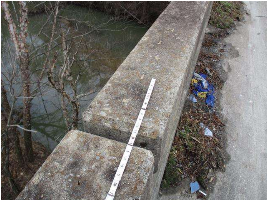
Span 3 Right Bridge Rail: UP TO 0.03" LONGITUDINAL AND VERTICAL CRACKS IN TOP AND ENDS OF RAIL IN VARIOUS LOCATIONS
