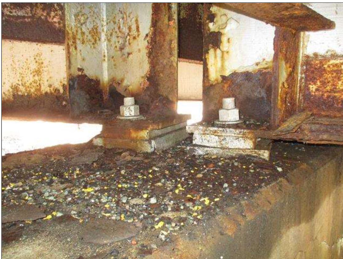
Span 2 Beam 3 - Far Bearing - Protective System: AREAS OF DETERIORATED PAINT SYSTEM THROUGHOUT BEAM 3 BEARING
