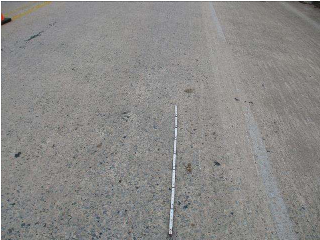
Span 4 Deck: SCALING WITH EXPOSED AGGREGATE IN TOP OF DECK THROUGHOUT TRAVEL LANES
