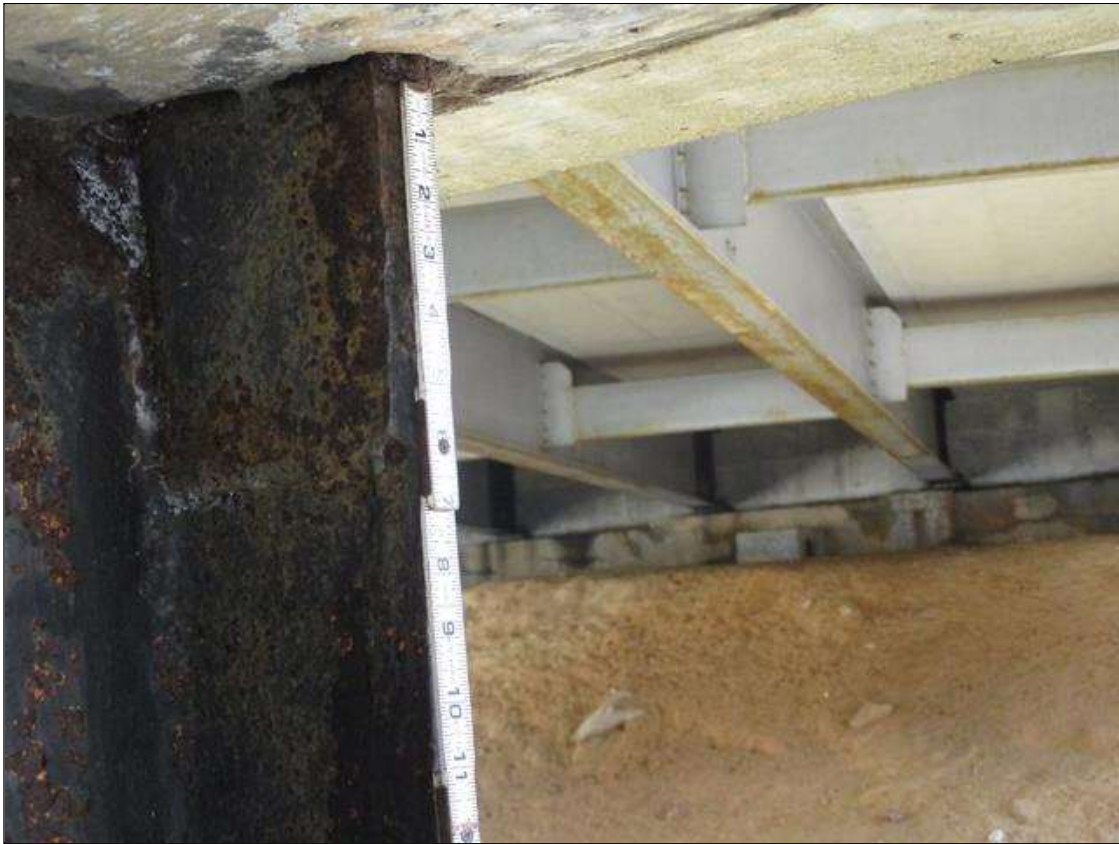
Bent 3 Pile 7: SURFACE CORROSION THROUGHOUT UP TO 12" WIDE X 9" HIGH PLATE REPAIR WELDED TO FACE OF FAR FLANGE AT BOTTOM OF CAP
