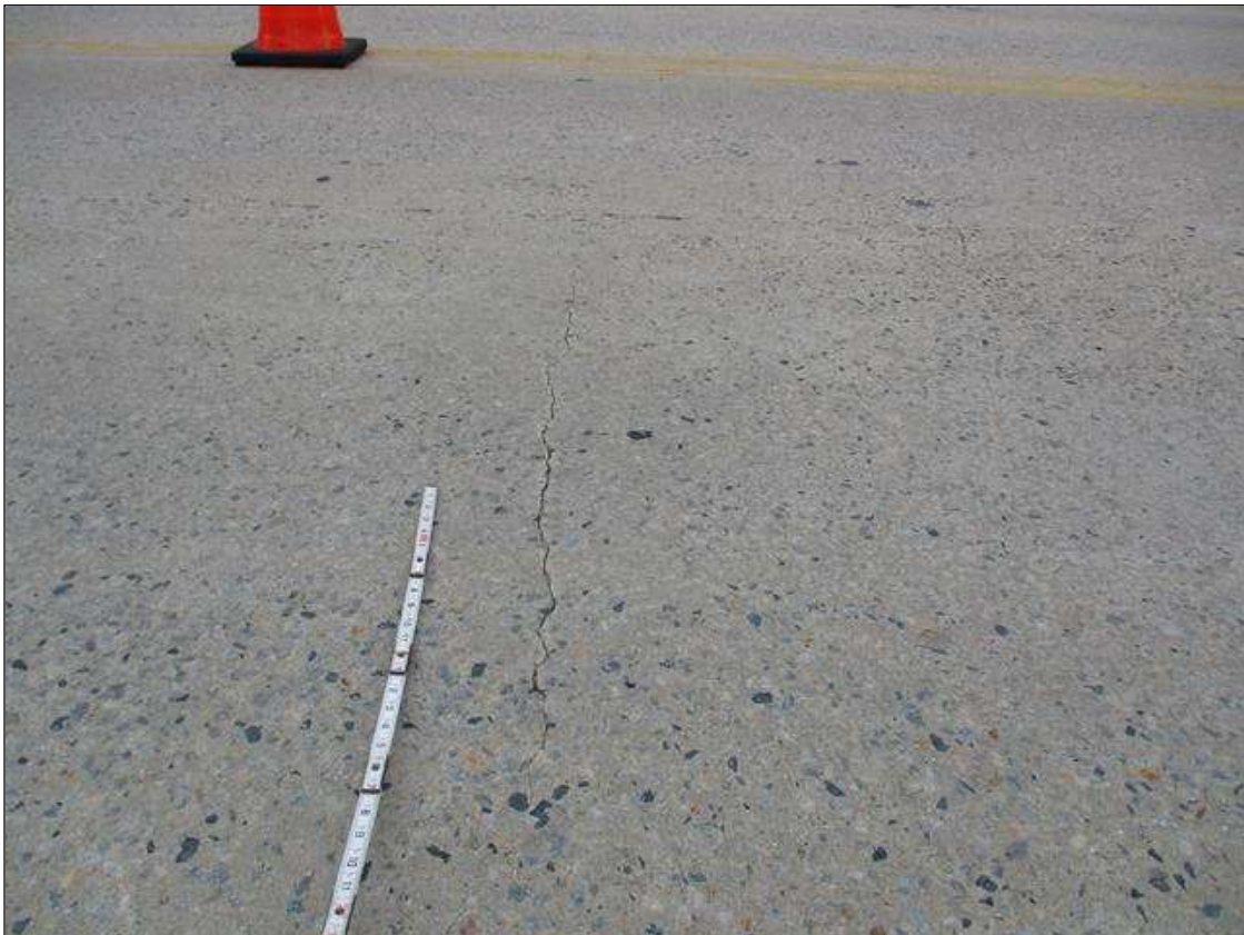
Span 2 Deck: UP TO 50" X 1/8" TRANSVERSE CRACKS IN TOP OF DECK IN EASTBOUND LANE AND RIGHT SHOULDER IN VARIOUS LOCATIONS
