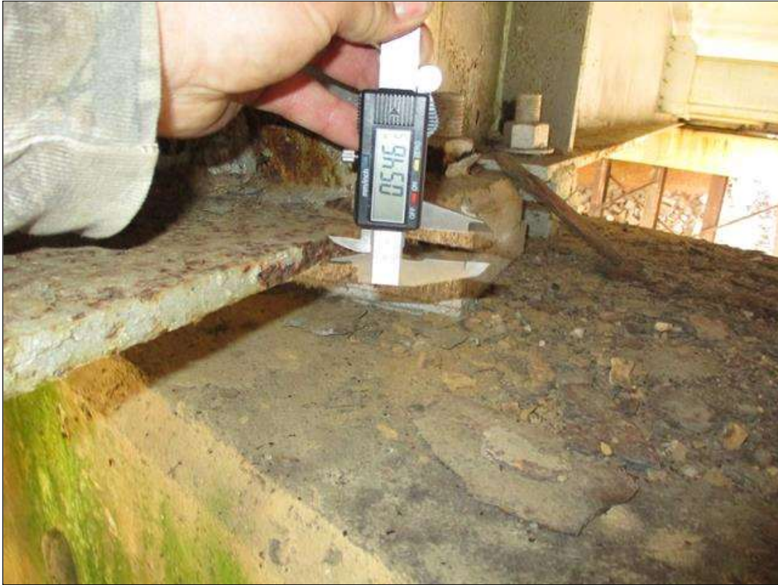
Span 2 Beam 5: (PAR) CORROSION ALONG BOTH FACES OF WEB AND BOTTOM FLANGE UP TO 17" LONG X 3" HIGH WITH NO MEASURABLE LOSS OF SECTION IN WEB, AND 14" LONG X 6" WIDE DOWN TO .546" RESIDUAL FLANGE AT BENT 2 BEARING
