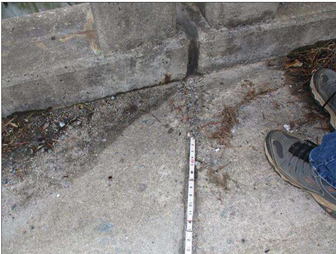
DIRT AND DEBRIS ACCUMULATION ALONG JOINT IN BOTH SHOULDERS (TYPICAL OF ALL JOINTS)
