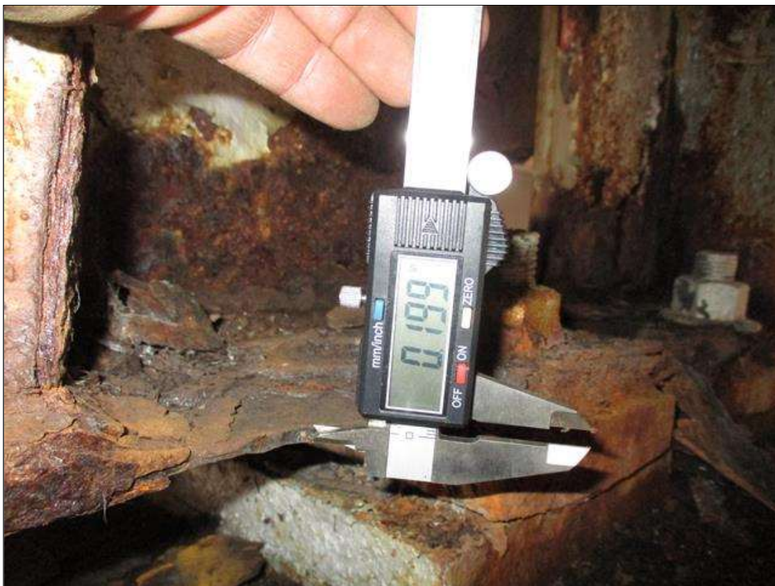
Span 3 Beam 3: (PAR) CORROSION ALONG BOTH FACES OF WEB AND BOTTOM FLANGE UP TO 15" LONG X 5" HIGH DOWN TO 0.503" RESIDUAL WEB, AND 18" LONG X 11 3/4" WIDE DOWN TO 0.199" RESIDUAL FLANGE AT BENT 3 BEARING
