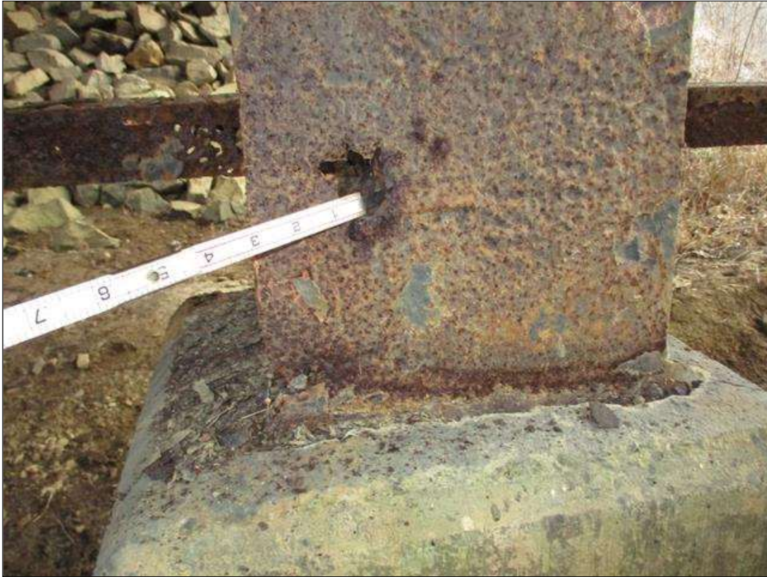
Bent 3 Pile 6: (PAR) CORROSION ALONG WEB AND BOTH FLANGES UP TO 19" HIGH X 11" WIDE WITH NO MEASURABLE LOSS OF SECTION IN WEB, AND 19" HIGH X 12" WIDE DOWN TO KNIFE'S EDGE RESIDUAL FLANGE WITH 2 LOCATIONS OF UP TO 6" HIGH X 3" WIDE 100% LOSS OF SECTION ABOVE CONCRETE ENCASEMENT
