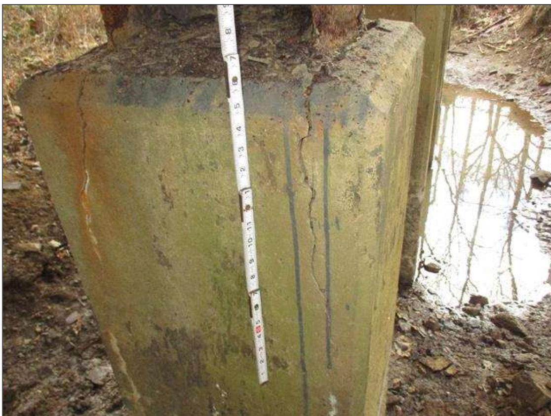
UP TO 1/4" TRANSVERSE AND VERTICAL CRACKS WITH AND WITHOUT EFFLORESCENCE IN ENCASEMENT
