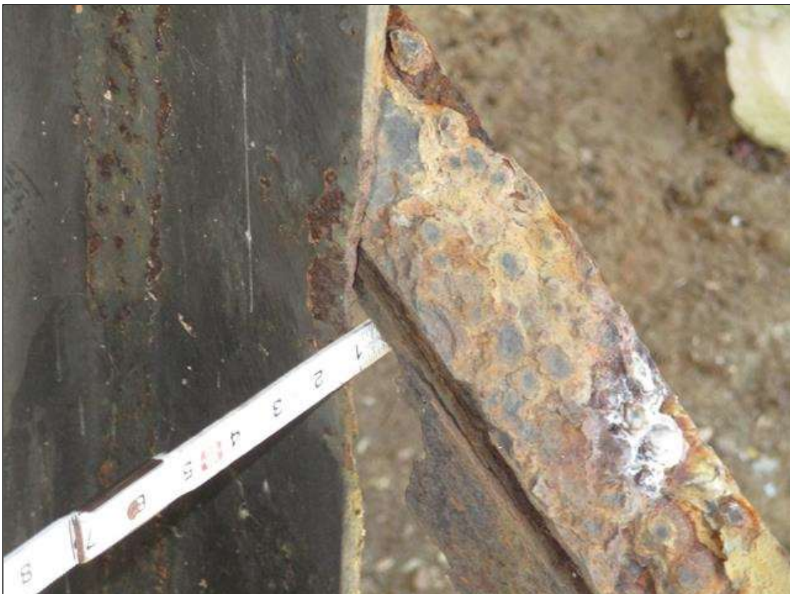
Bent 3 Pile 6: (PAR) CORROSION ALONG FAR FLANGE UP TO 5" HIGH X 12" WIDE DOWN TO 3/16" RESIDUAL FLANGE, APPROXIMATELY 4' FROM BOTTOM OF CAP
