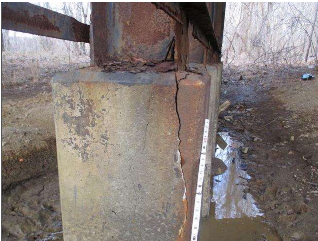
UP TO 1/4" TRANSVERSE & VERTICAL CRACKS WITH & WITHOUT EFFLORESCENCE IN ENCASEMENT. TOP 2' OF EAST FACE BEGINNING TO DELAMINATE
