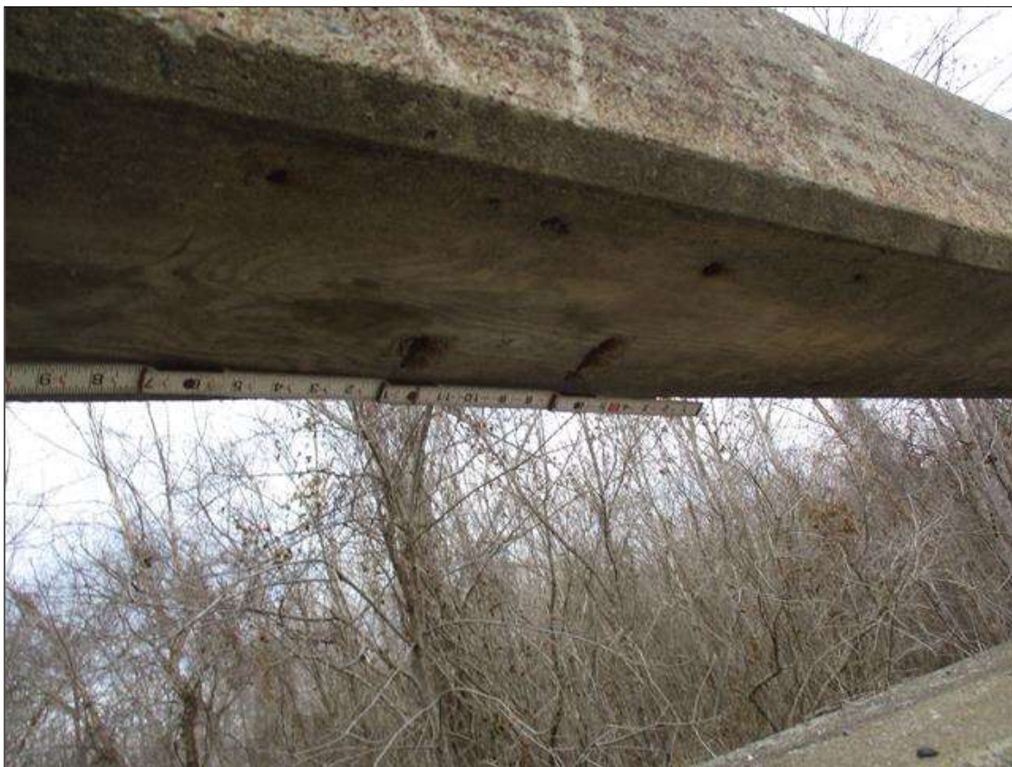
Span 3 Left Bridge Rail: WITHIN 8' OF BENT 3 JOINT, (3) 3" DIAMETER X 0.25" DEEP SPALLS WITH EXPOSED REBAR UNDER RAILING
