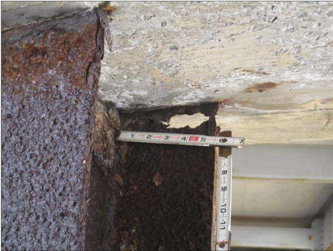
Bent 3 Pile 5: (PAR) CORROSION ALONG BOTH FLANGES UP TO 24" HIGH X 12" WIDE, 100% SECTION LOSS ON FLANGE WITH UP TO 2 1/2" WIDE X 1" HIGH HOLES AT BOTTOM OF CAP
