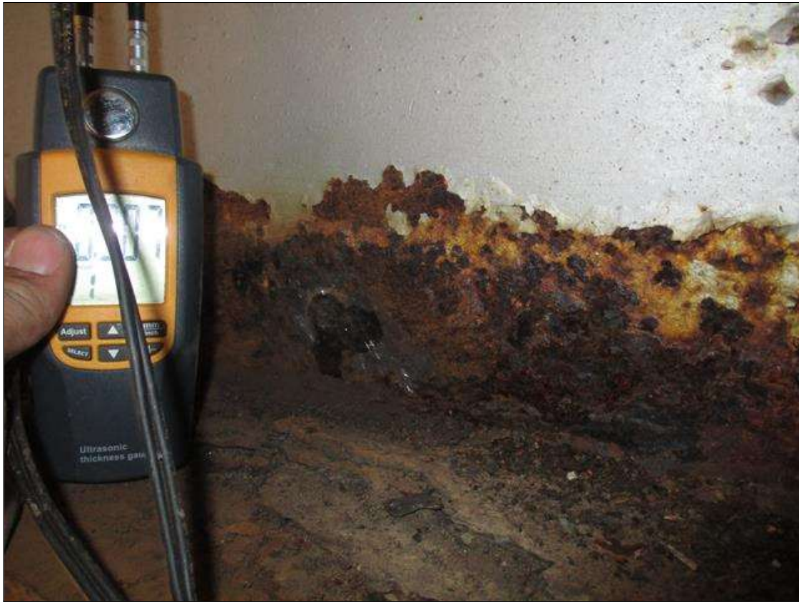
Span 1 Beam 2: (PAR) CORROSION ALONG RIGHT FACE OF WEB AND BOTTOM FLANGE UP TO 39" LONG X 10" HIGH DOWN TO 0.3" RESIDUAL WEB, AND 35" LONG X 5" WIDE DOWN TO 0.48" RESIDUAL FLANGE AT BENT 1 BEARING
