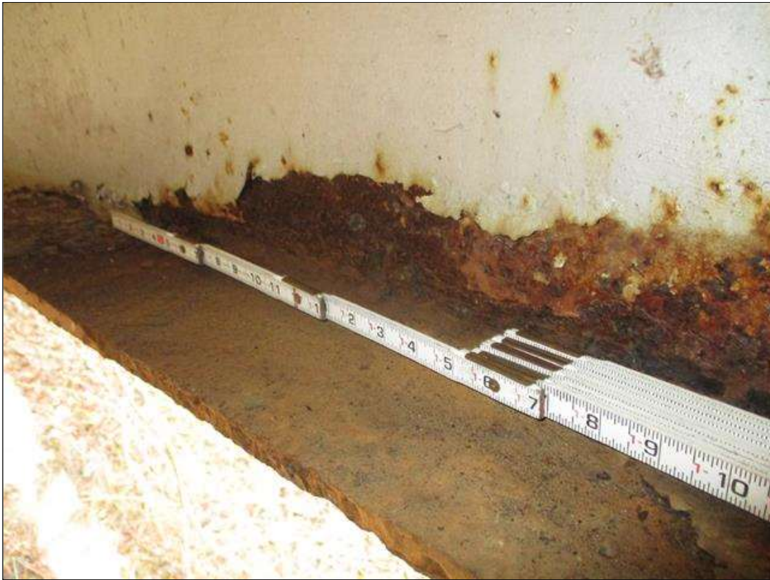
TYPICAL CORROSION IN SPAN 1, BEAM 1 @ BENT 1
