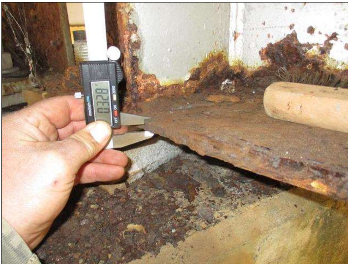
Span 2 Beam 2: (PAR) CORROSION ALONG BOTH FACES OF WEB AND BOTTOM FLANGE UP TO 33" LONG X 6" HIGH DOWN TO 0.275" RESIDUAL WEB, AND 34" LONG X 5" WIDE DOWN TO .328" RESIDUAL FLANGE AT BENT 2 BEARING
