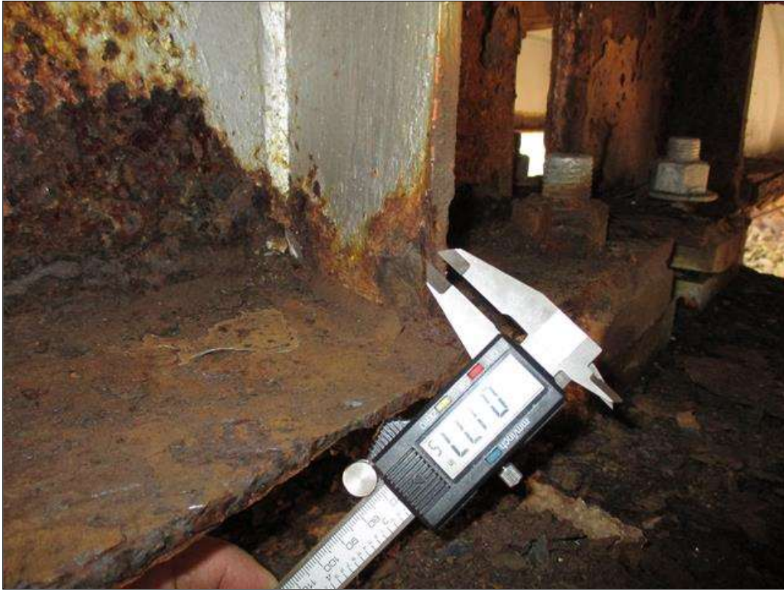
Span 2 Beam 3: (PAR) CORROSION ALONG BOTH FACES OF WEB AND BOTTOM FLANGE UP TO 25" LONG X 24" HIGH DOWN TO RESIDUAL WEB WITH 3" X 3" LOSS OF SECTION, AND 24" LONG X 11 3/4" WIDE DOWN TO .177" RESIDUAL FLANGE AT BENT 2 BEARING
