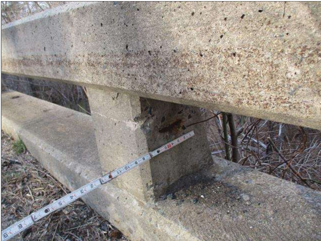
Span 4 Left Bridge Rail: 4 1/2" X 2 1/2" X 1/4" DEEP SPALL WITH EXPOSED REBAR IN EAST FACE OF RAIL POST NEAR MIDSPAN
