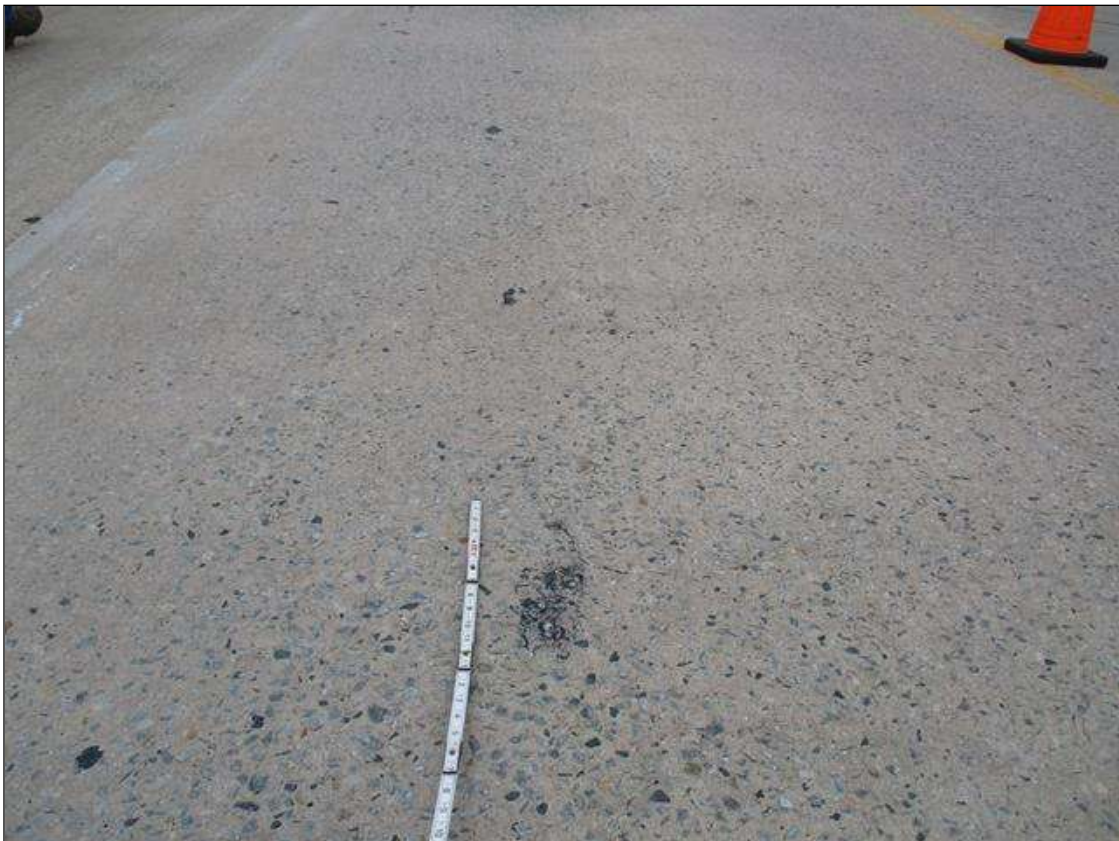
Span 2 Deck: 1320 SF OF SCALING WITH EXPOSED AGGREGATE IN TOP OF DECK THROUGHOUT TRAVEL LANES
