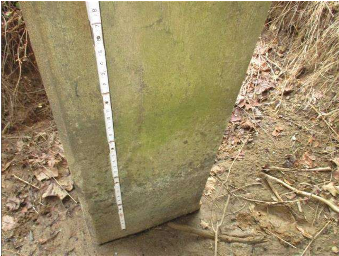
UP TO 0.03" TRANSVERSE & VERTICAL CRACKS IN ENCASEMENT
