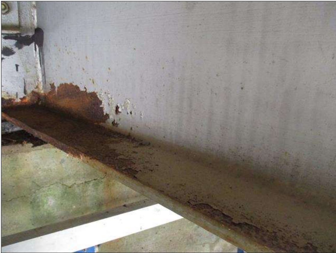
TYPICAL DETERIORATED PAINT SYSTEM (SPAN 3, BEAM 5)
