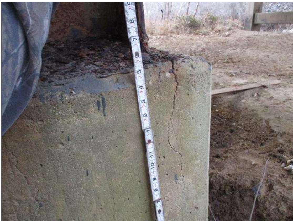
UP TO 1/16" TRANSVERSE & VERTICAL CRACKS IN ENCASEMEN (BENT 3, PILE 4)
