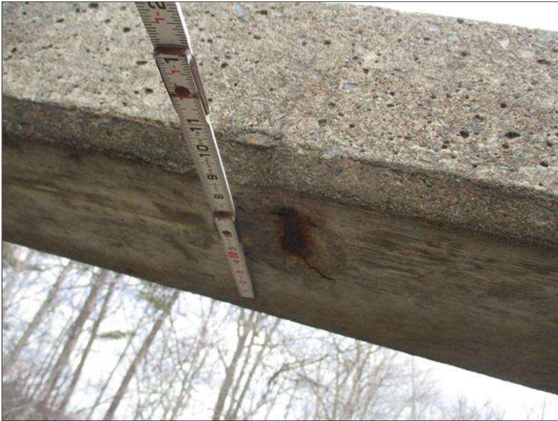
Span 1 Left Bridge Rail: 14 SPALLS WITH EXPOSED REBAR UP TO 6" X 4" X 3/4" DEEP IN BOTTOM OF RAIL IN VARIOUS LOCATIONS
