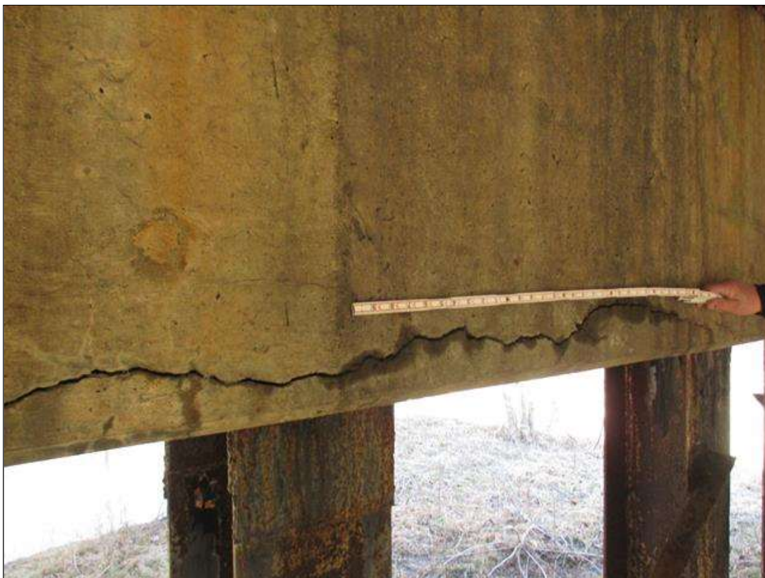
Bent 3 Cap 1: UP TO 1/4" LONGITUDINAL AND HORIZONTAL CRACKS AND HAIRLINE MAP CRACKING WITH AND WITHOUT EFFLORESCENCE IN BOTTOM AND BOTH FACES OF CAP
