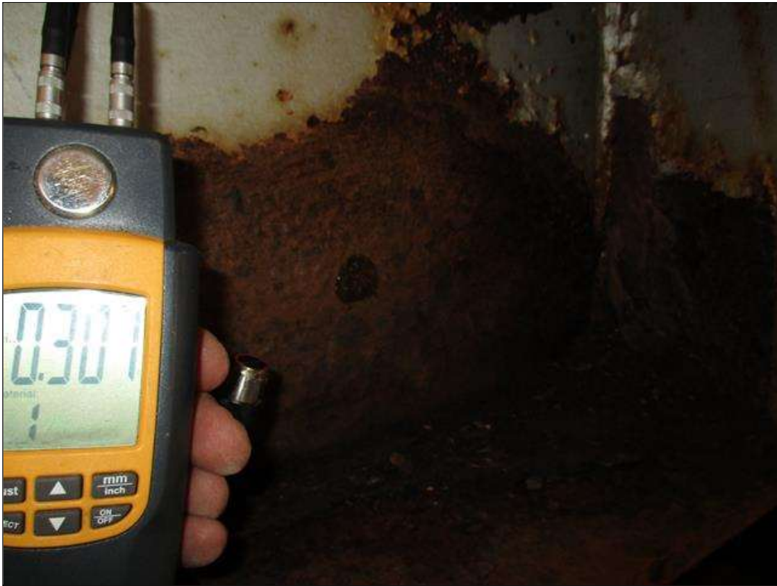
Span 3 Beam 5: (PAR) CORROSION ALONG BOTH FACES OF WEB AND BOTTOM FLANGE UP TO 24" LONG X 13" HIGH DOWN TO 0.301" RESIDUAL WEB, AND 29" LONG X 11 3/4" WIDE DOWN TO .443" RESIDUAL FLANGE AT BENT 3 BEARING
