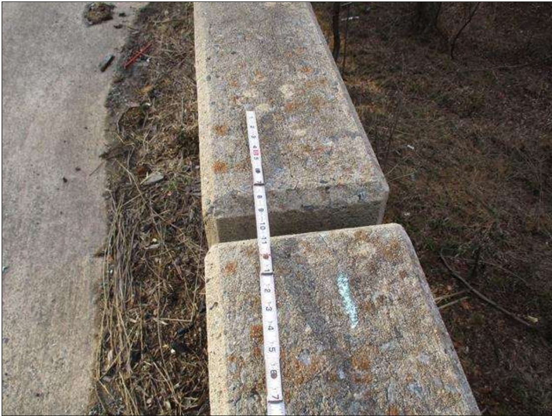
Span 4 Left Bridge Rail: UP TO 0.03" LONGITUDINAL AND VERTICAL CRACKS IN TOP AND ENDS OF RAIL IN VARIOUS LOCATIONS
