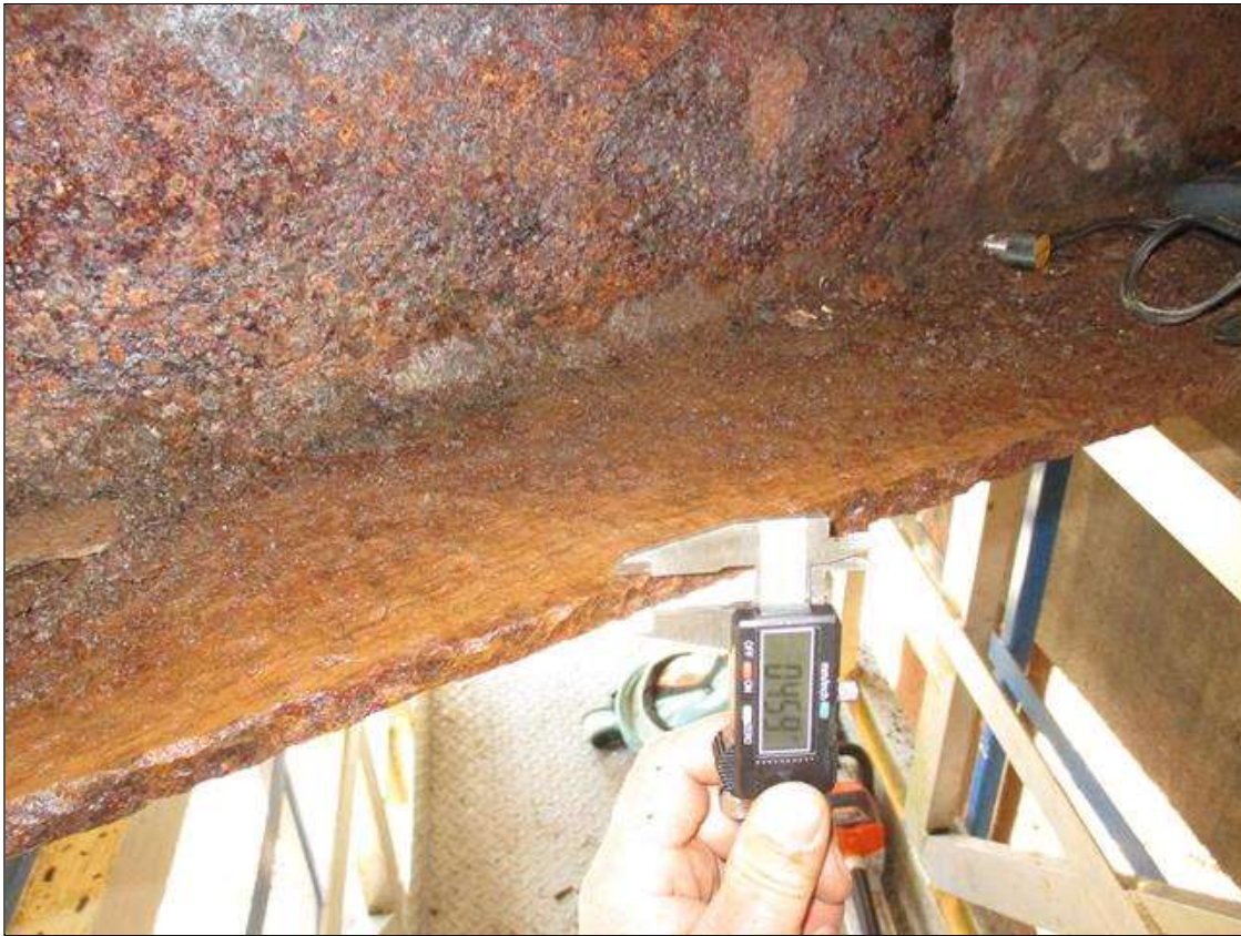
Span 4 Beam 5: (PAR) CORROSION ALONG BOTH FACES OF WEB AND BOTTOM FLANGE UP TO 105" LONG X 19" HIGH DOWN TO 0.358" RESIDUAL WEB, AND 72" LONG X 11 3/4" WIDE DOWN TO 0.459" RESIDUAL FLANGE AT BENT 3 BEARING
