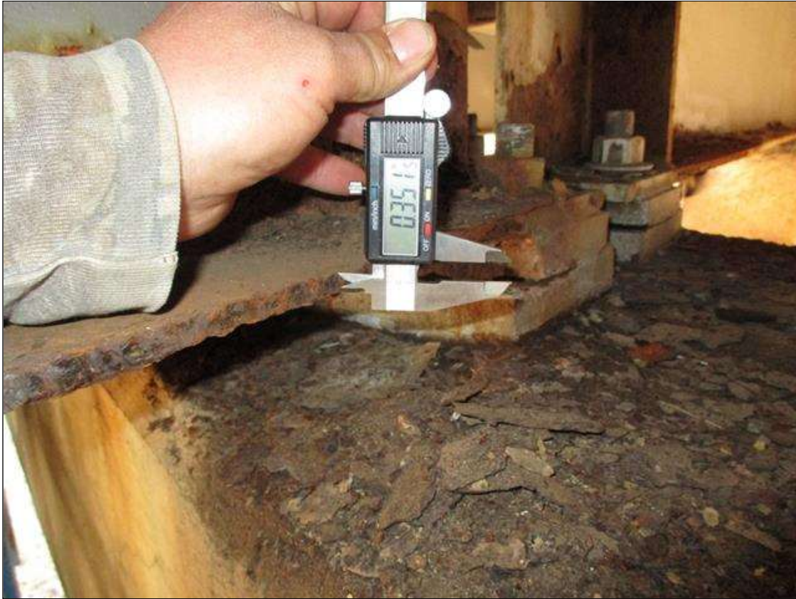
Span 3 Beam 2: (PAR) CORROSION ALONG BOTH FACES OF WEB AND BOTTOM FLANGE UP TO 32" LONG X 5" HIGH DOWN TO 0.212" RESIDUAL WEB, AND 34" LONG X 11 3/4" WIDE DOWN TO 0.350" RESIDUAL FLANGE AT BENT 3 BEARING
