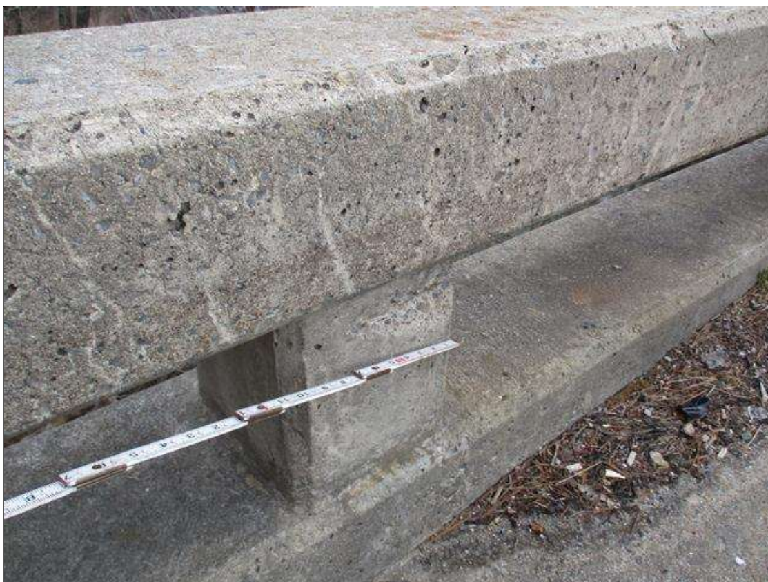
Span 1 Left Bridge Rail: THREE (3) SPALLS UP TO 6" X 3" X 1/2" DEEP IN FACE OF RAIL POSTS IN VARIOUS LOCATIONS
