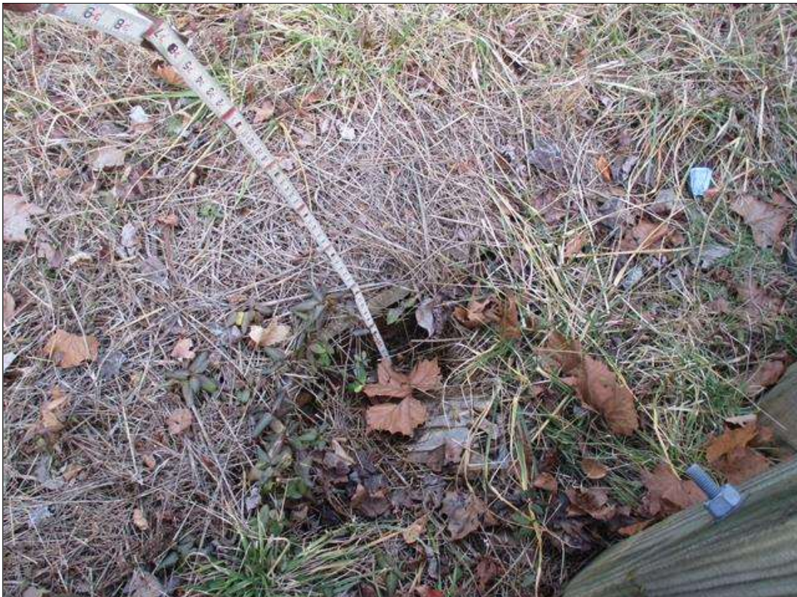
(PAR) BRIDGE DRAINAGE, CLOGGED EITHER PARTIALLY OF FULLY WITH VEGETATION GROWTH. (16) ALONG RIGHT CURB & (5) ALONG LEFT CURB
