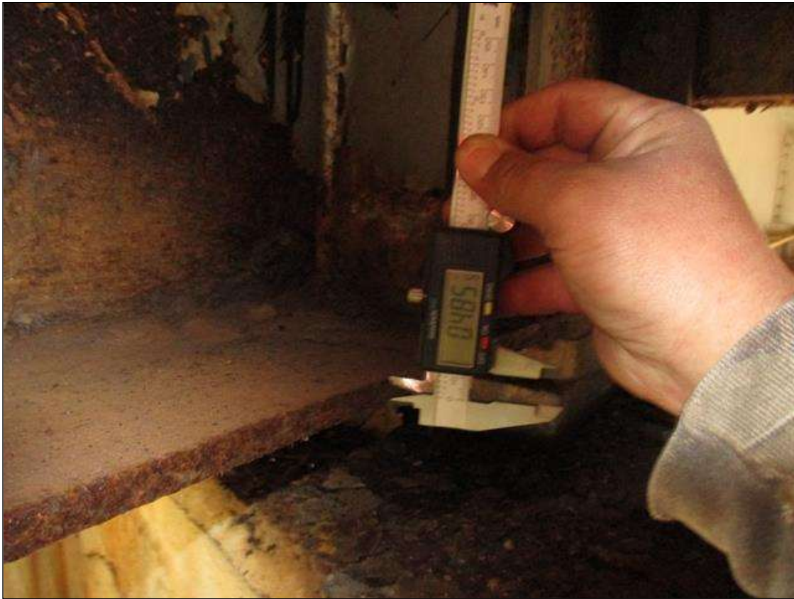
Span 3 Beam 4: (PAR) CORROSION ALONG BOTH FACES OF WEB AND BOTTOM FLANGE UP TO 38" LONG X 7" HIGH DOWN TO 0.413" RESIDUAL WEB, AND 41" LONG X 11 3/4" WIDE DOWN TO 0.485" RESIDUAL FLANGE AT BENT 3 BEARING
