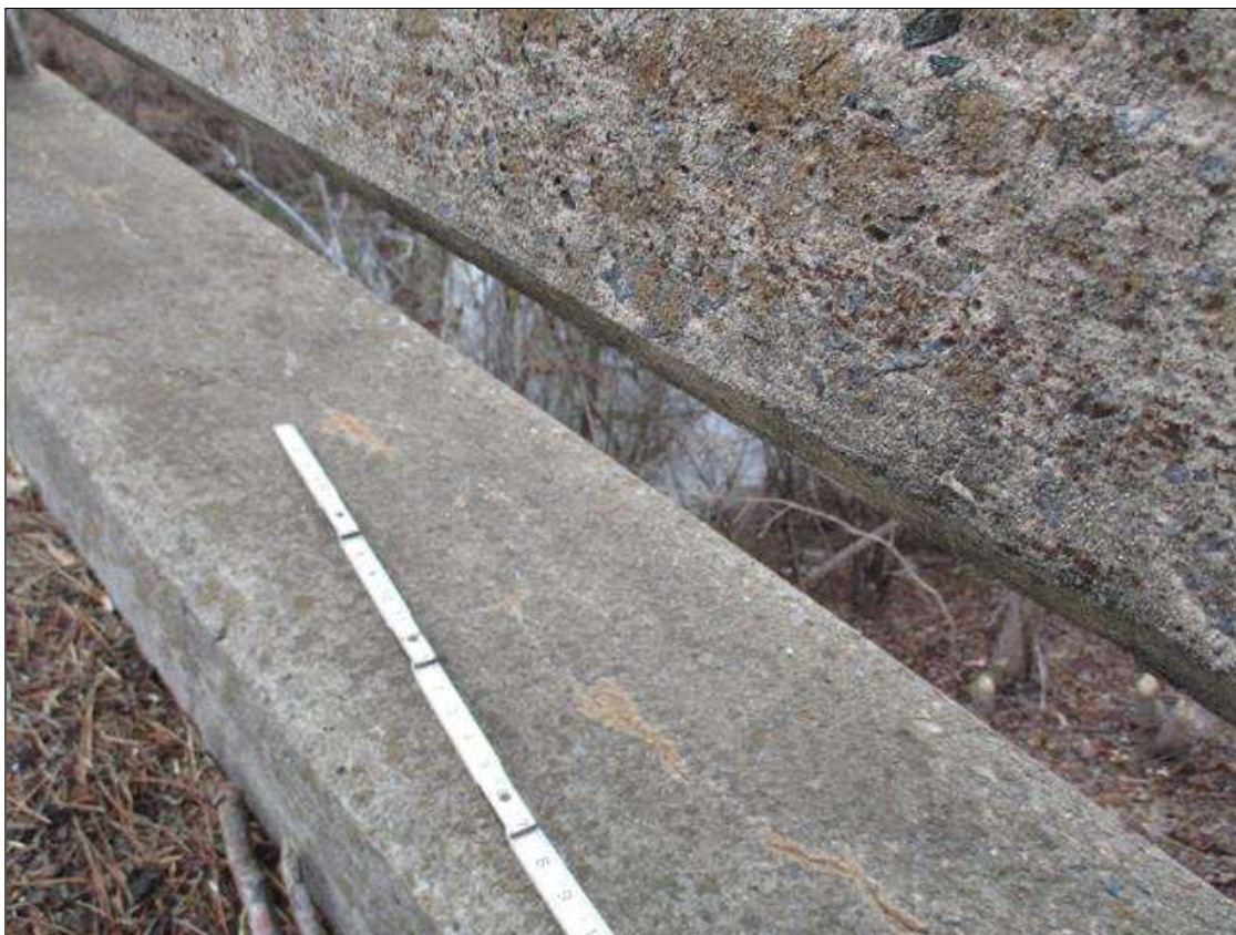
Span 1 Right Bridge Rail: UP TO 0.05" LONGITUDINAL, TRANSVERSE, VERTICAL AND MAP CRACKS IN TOP AND FACES OF RAIL IN VARIOUS LOCATIONS
