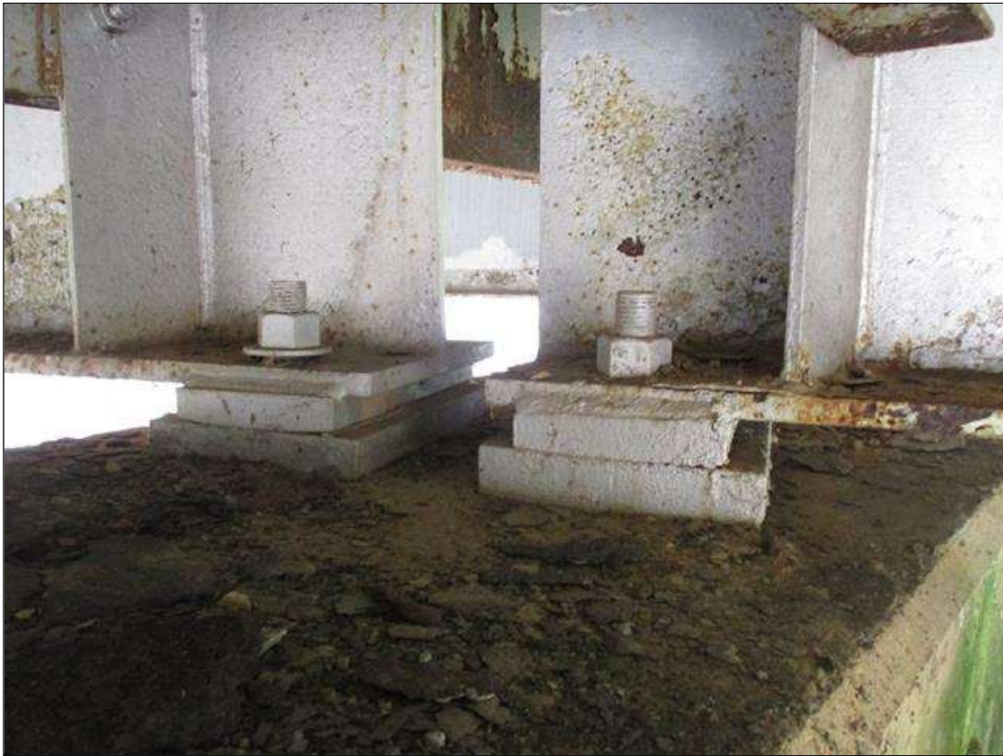
Span 2 Beam 4 - Far Bearing - Protective System: AREAS OF DETERIORATED PAINT SYSTEM THROUGHOUT BEAM 4 BEARING
