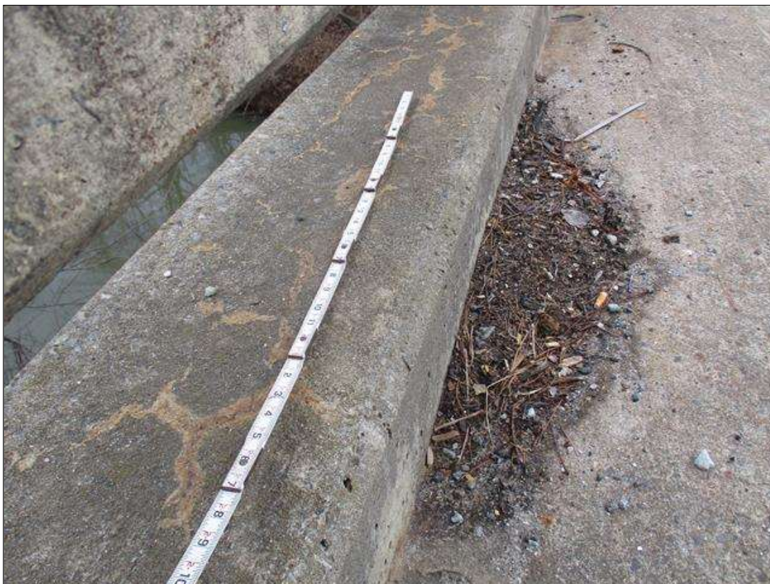
Span 2 Left Bridge Rail: ON TOP OF CURB THROUGHOUT, LESS THAN 0.01" WIDE CRACKING WITH EFFLORESCENCE
