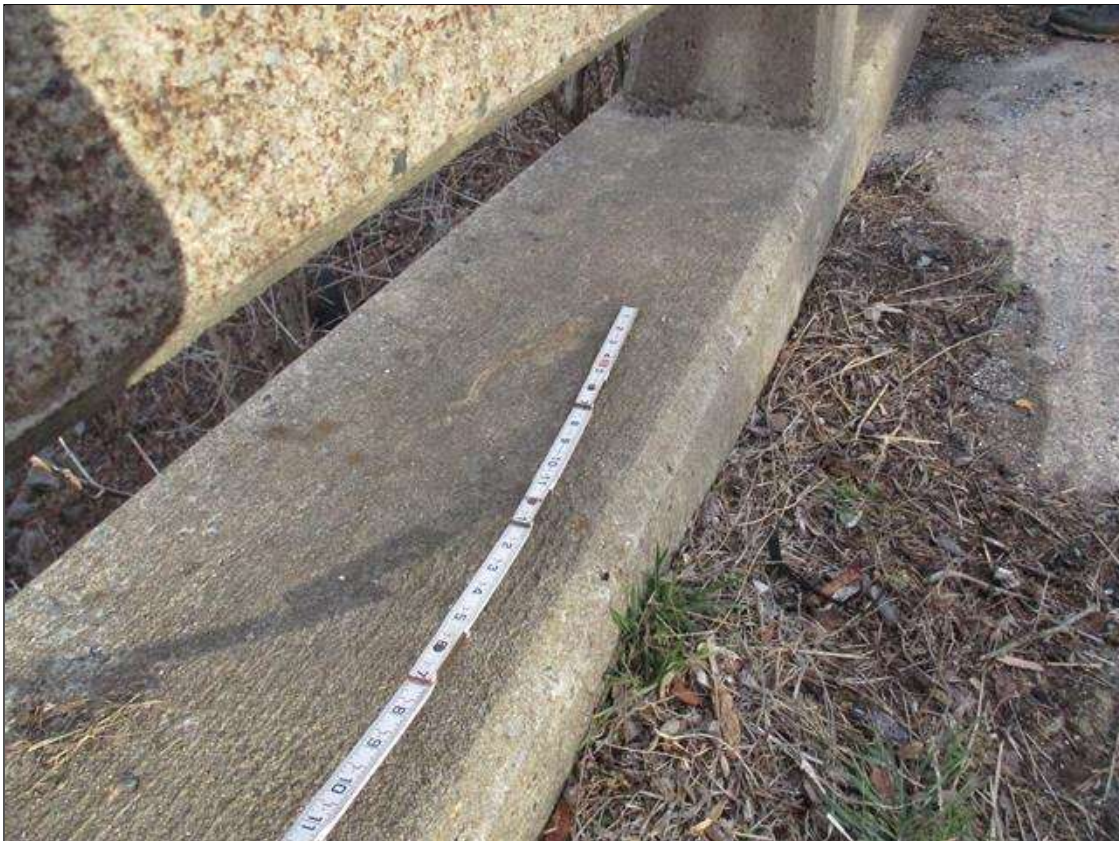
Span 4 Left Bridge Rail: ON TOP OF CURB THROUGHOUT, LESS THAN 0.01" WIDE CRACKING WITH EFFLORESCENCE
