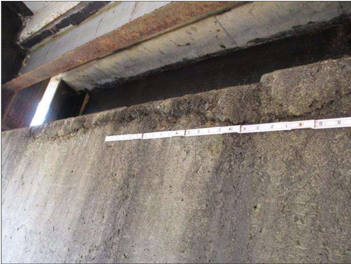
Bent 3 Cap 1: UP TO 1/4" LONGITUDINAL AND HORIZONTAL CRACKS AND HAIRLINE MAP CRACKING WITH AND WITHOUT EFFLORESCENCE IN BOTTOM AND BOTH FACES OF CAP
