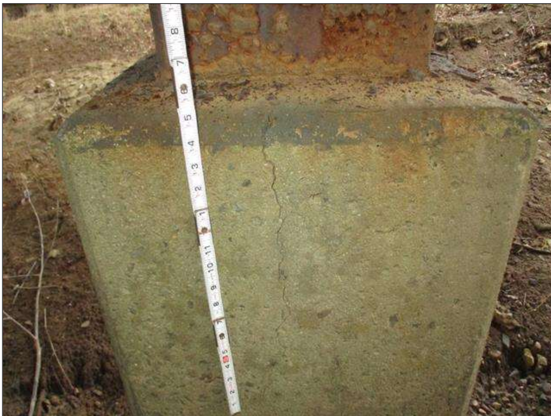
UP TO 1/16" TRANSVERSE & VERTICAL CRACKS IN ENCASEMEN (BENT 3, PILE 3)
