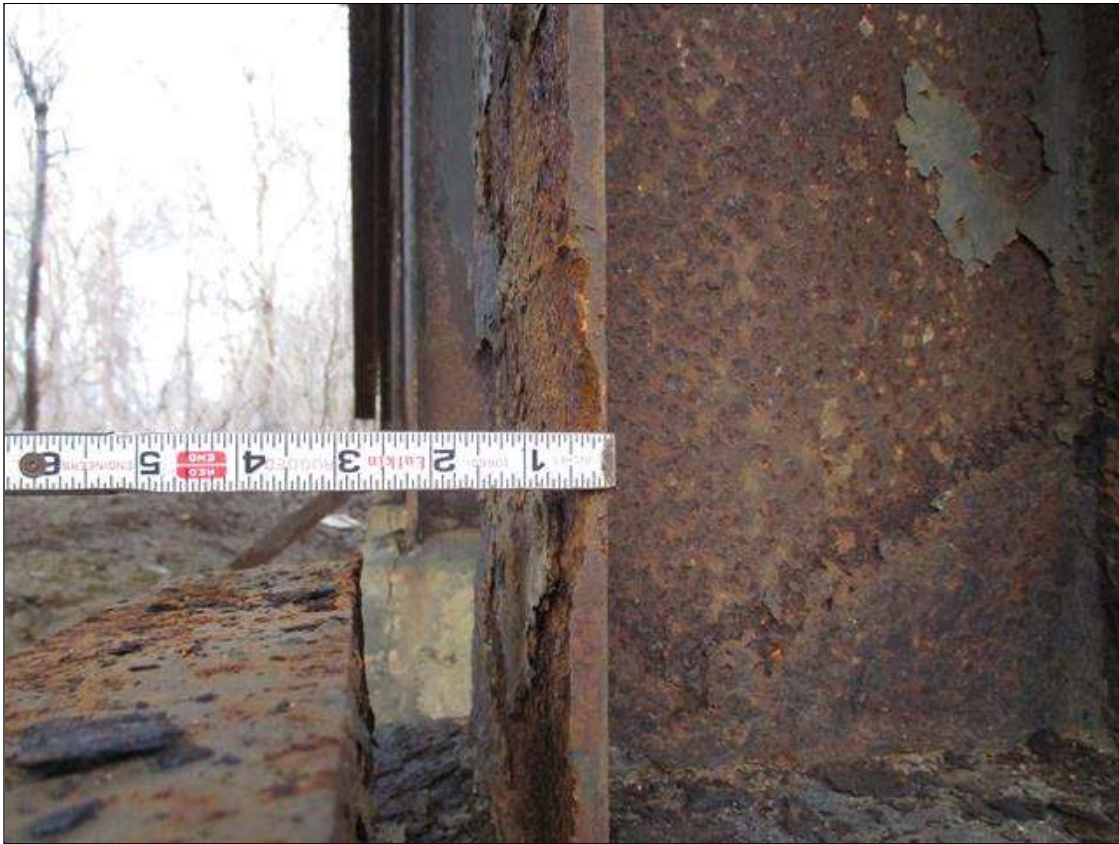
Bent 3 Pile 7: (PAR) CORROSION ALONG BOTH FLANGES UP TO 17" HIGH X 12" WIDE DOWN TO 1/4" RESIDUAL FLANGE ABOVE CONCRETE ENCASEMENT
