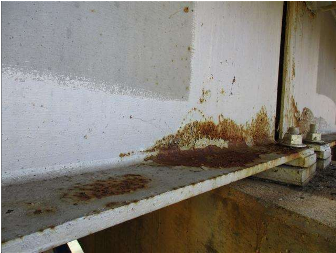
Span 1 Beam 6: AREAS OF SURFACE CORROSION THROUGHOUT WEB AND BOTH FLANGES IN VARIOUS LOCATIONS
