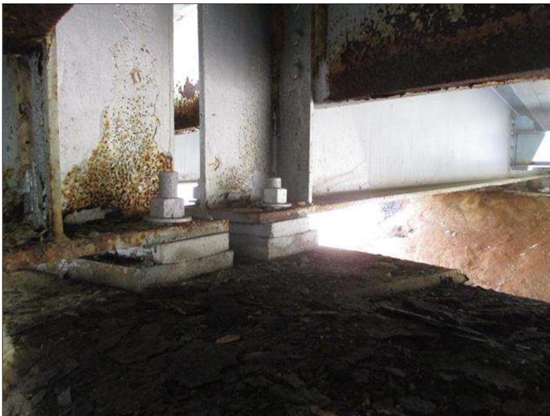
Span 2 Beam 3 - Near Bearing - Protective System: AREAS OF DETERIORATED PAINT SYSTEM THROUGHOUT BEAM 3 BEARING
