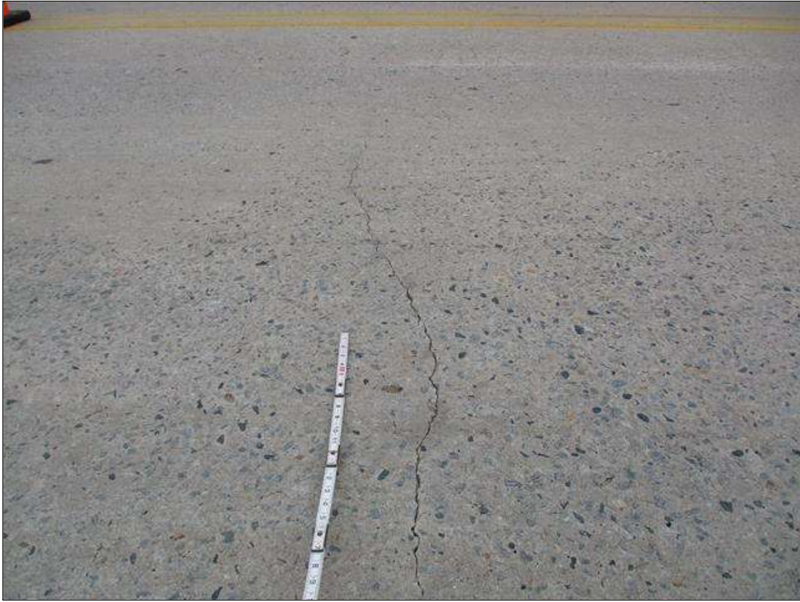
Span 3 Deck: UP TO 0.02" MAP CRACKS IN TOP OF DECK IN VARIOUS LOCATIONS
