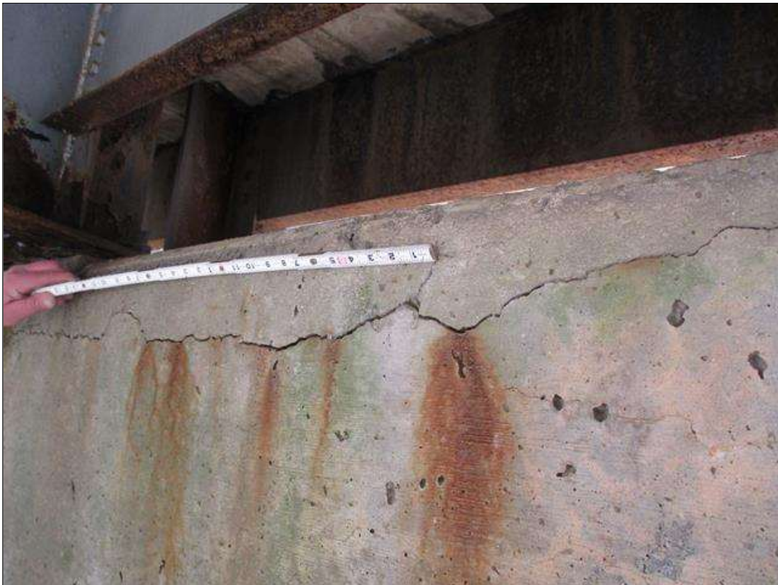
Bent 3 Cap 1: UP TO 1/4" LONGITUDINAL AND HORIZONTAL CRACKS AND HAIRLINE MAP CRACKING WITH AND WITHOUT EFFLORESCENCE IN BOTTOM AND BOTH FACES OF CAP
