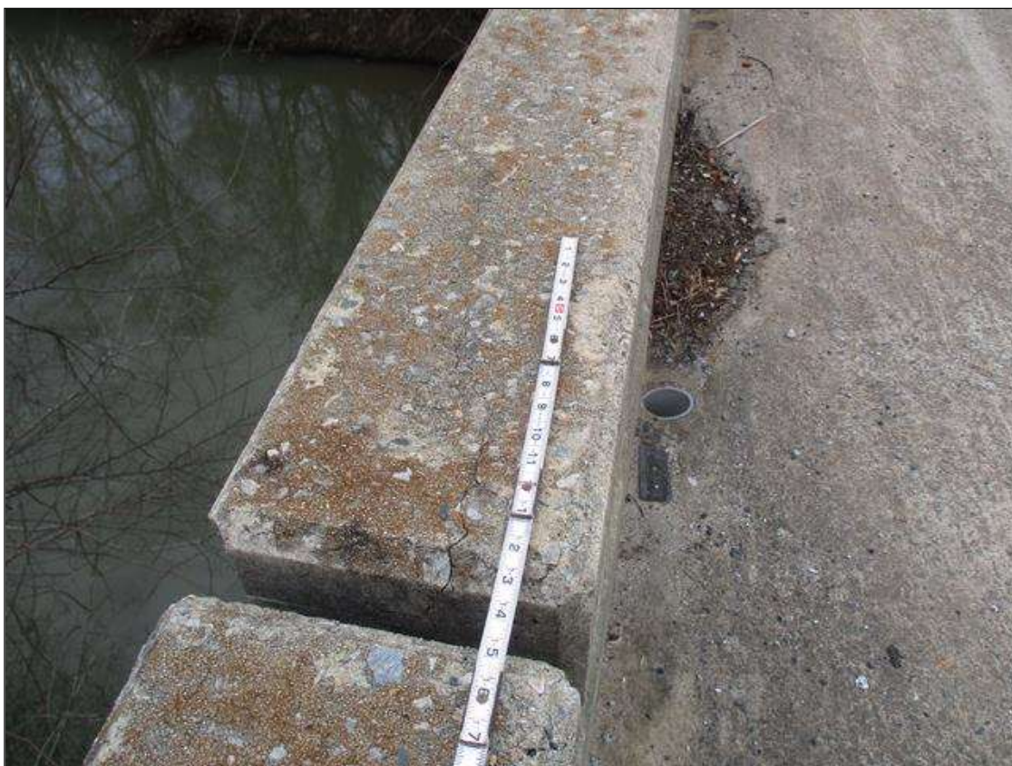
Span 2 Left Bridge Rail: UP TO 0.035" LONGITUDINAL AND VERTICAL CRACKS IN TOP AND ENDS OF RAIL IN VARIOUS LOCATIONS
