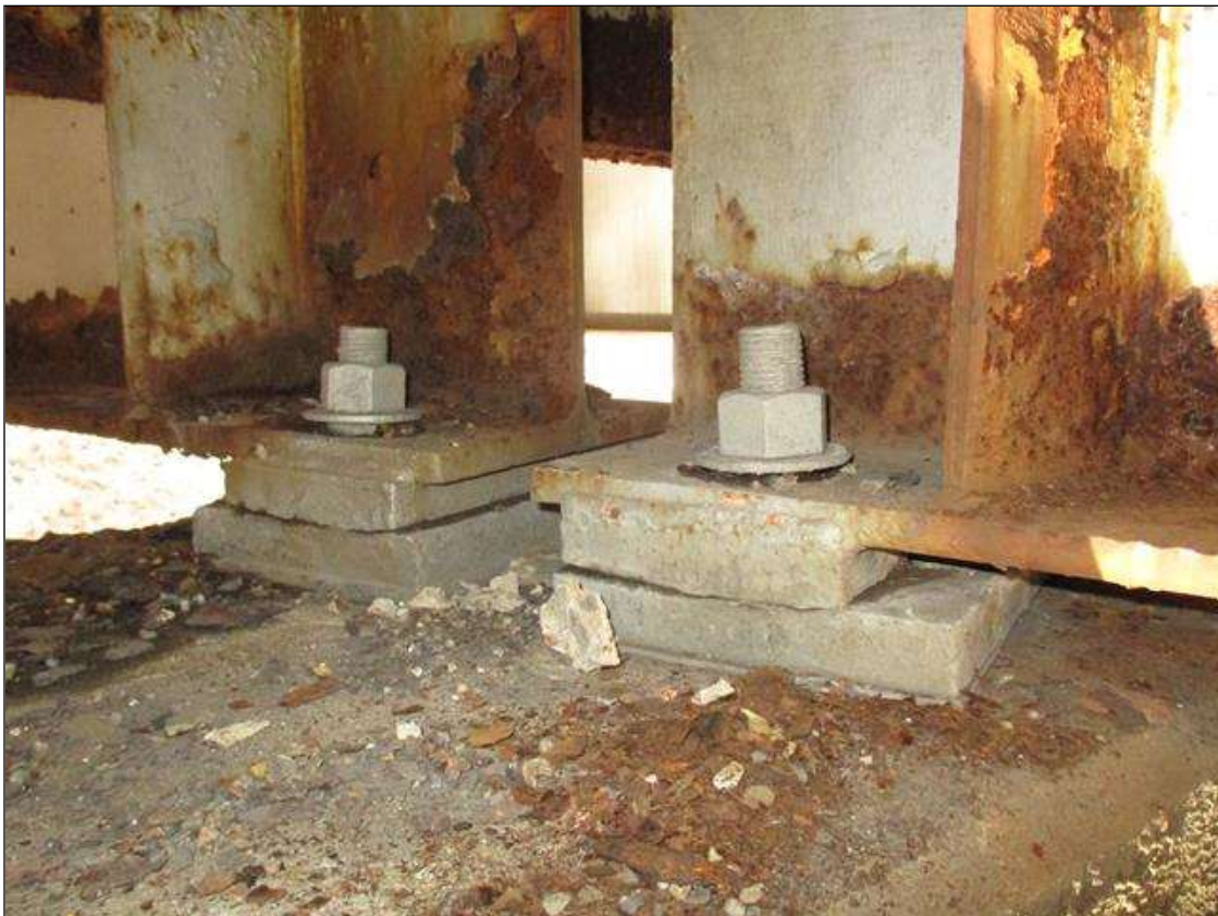
Span 1 Near Bearing: SURFACE CORROSION THROUGHOUT BEAM 1 BEARING
