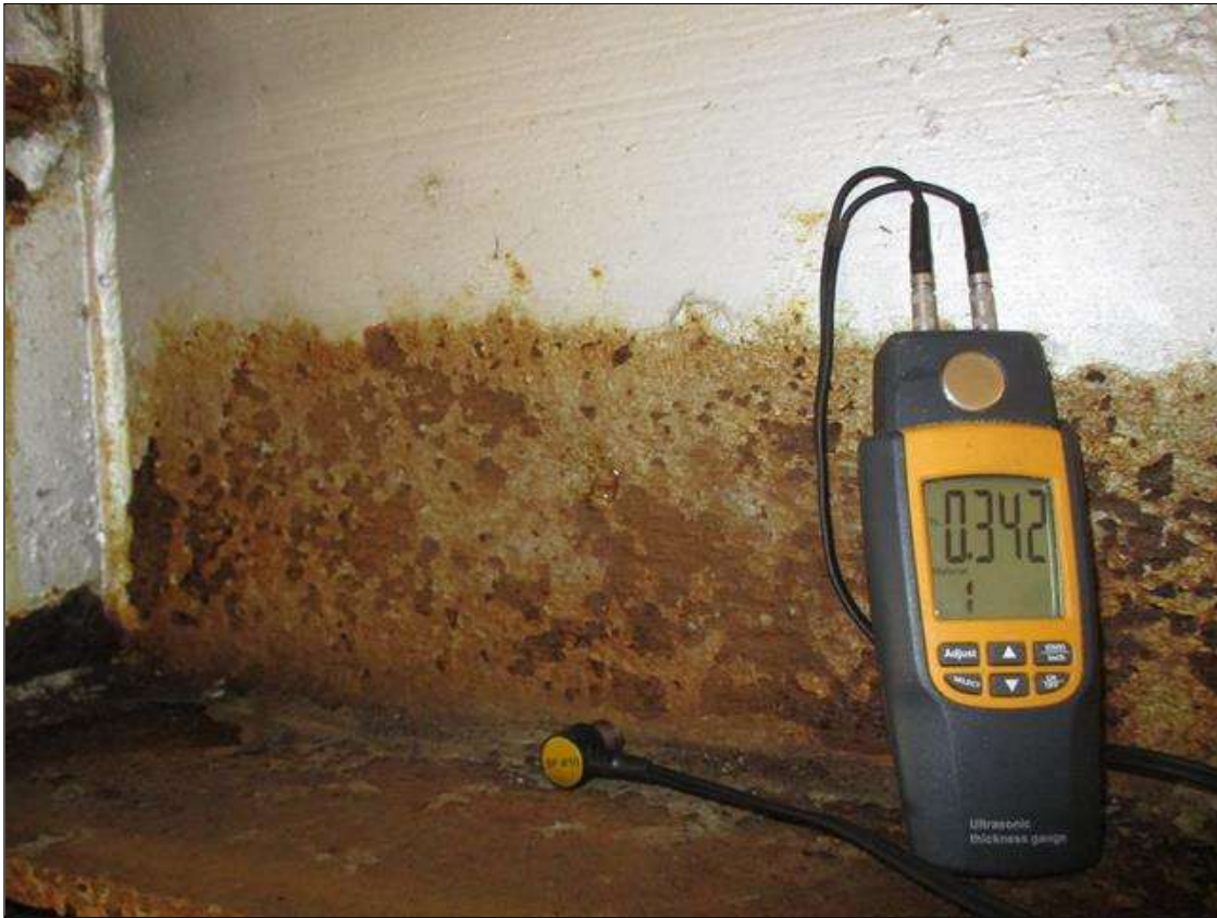
Span 3 Beam 4: (PAR) CORROSION ALONG BOTH FACES OF WEB AND BOTTOM FLANGE UP TO 58" LONG X 6" HIGH DOWN TO 0.342" RESIDUAL WEB, AND 39" LONG X 11 3/4" WIDE DOWN TO 0.505" RESIDUAL FLANGE AT BENT 2 BEARING
