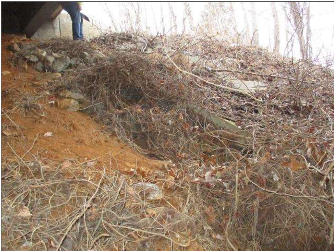
CONCRETE SWALE @ END BENT 1 ON LEFT SIDE IS UNDERMINED FOR ITS ENTIRE LENGTH
