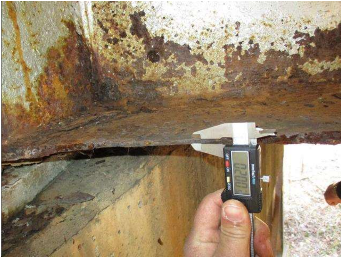
Span 4 Beam 3: (PAR) CORROSION ALONG BOTH FACES OF WEB AND BOTTOM FLANGE UP TO 14" LONG X 8" HIGH DOWN TO 0.236" RESIDUAL WEB, AND 24" LONG X 11 3/4" WIDE DOWN TO 0.200" RESIDUAL FLANGE AT BENT 3 BEARING
