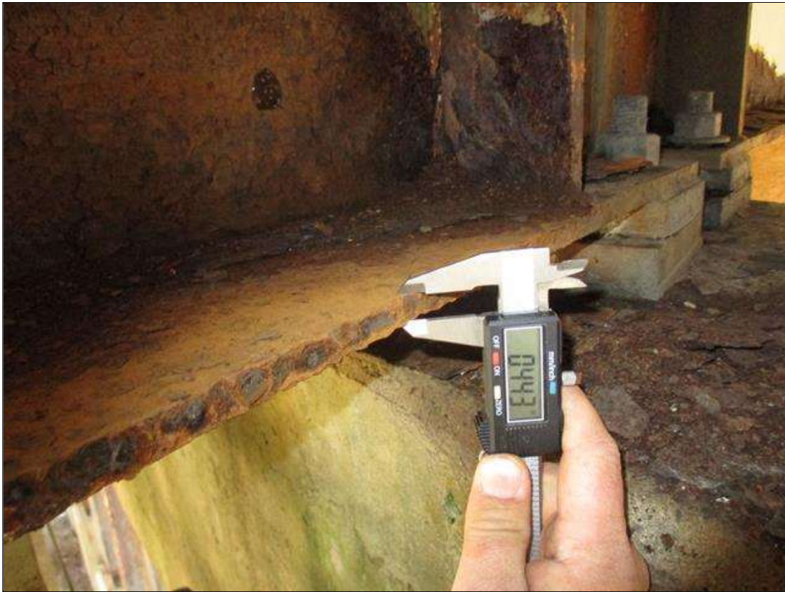
Span 3 Beam 5: (PAR) CORROSION ALONG BOTH FACES OF WEB AND BOTTOM FLANGE UP TO 24" LONG X 13" HIGH DOWN TO 0.301" RESIDUAL WEB, AND 29" LONG X 11 3/4" WIDE DOWN TO .443" RESIDUAL FLANGE AT BENT 3 BEARING
