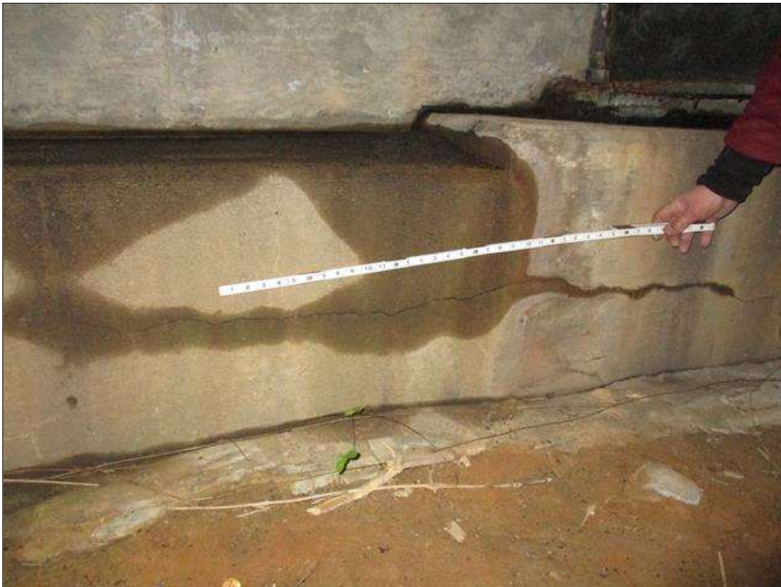
End Bent 2 Cap 1: UP TO 5/16" LONGITUDINAL AND HORIZONTAL CRACKS IN FACE OF CAP BENEATH BAYS 4 AND 5
