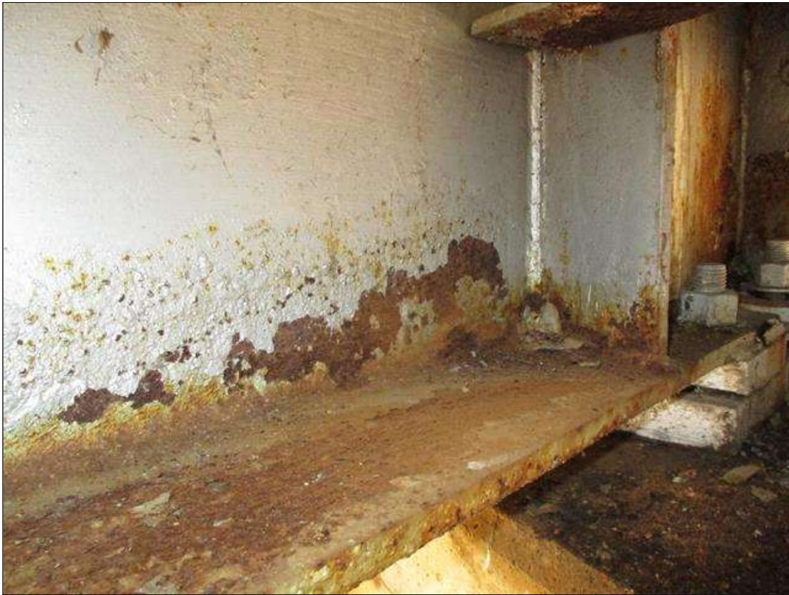
TYPICAL SURFACE CORROSION (SPAN 2, BEAM 4)
