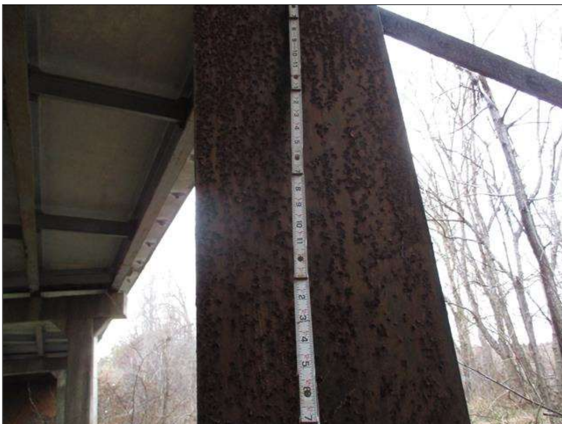
TYPICAL SURFACE CORROSION & DETERIORATED PAINT SYSTEM (BENT 3, PILE 2)
