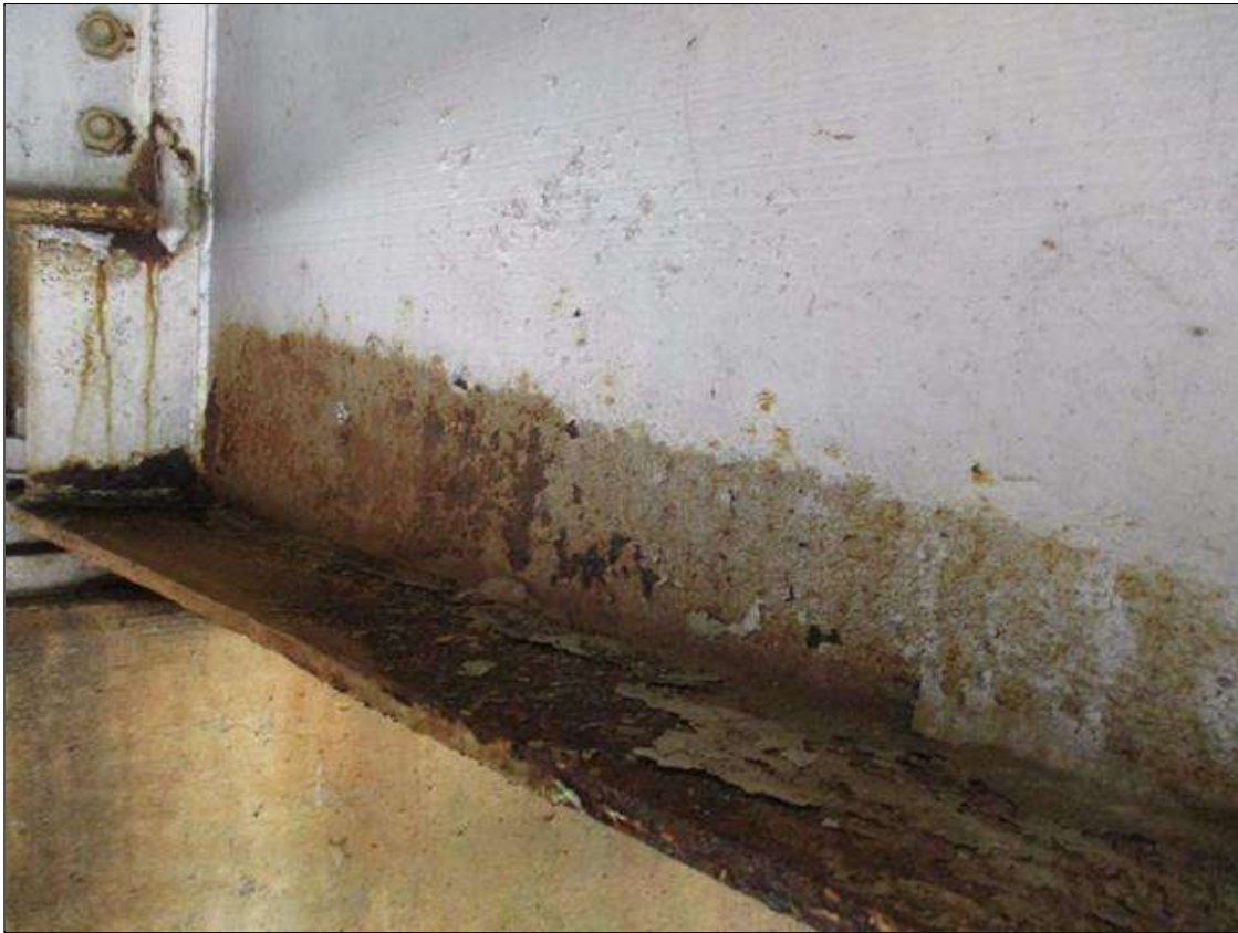
TYPICAL DETERIORATED PAINT SYSTEM (SPAN 3, BEAM 4)
