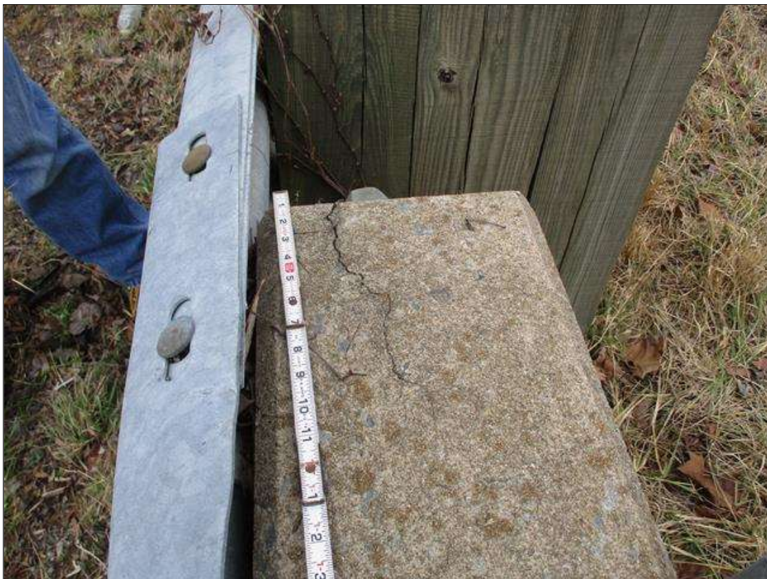
Span 4 Right Bridge Rail: AT END BENT 2 END RAIL, 1' LONG X UP TO 0.0625" WIDE ALONG TOP OF RAIL
