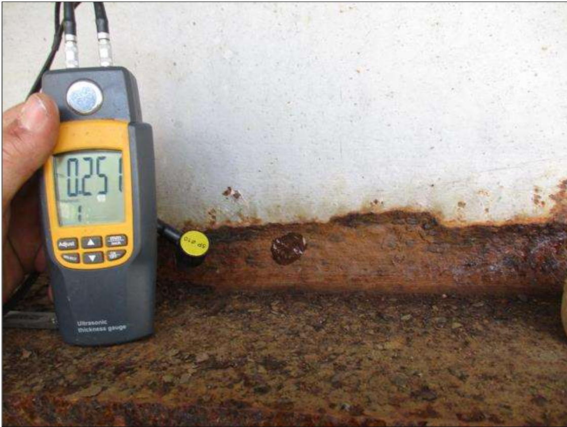
Span 3 Beam 1: (PAR) CORROSION EXTENDING 5' FROM BENT 2 WEB, 0.251" REMAINING UP 3" FROM FLANGE
