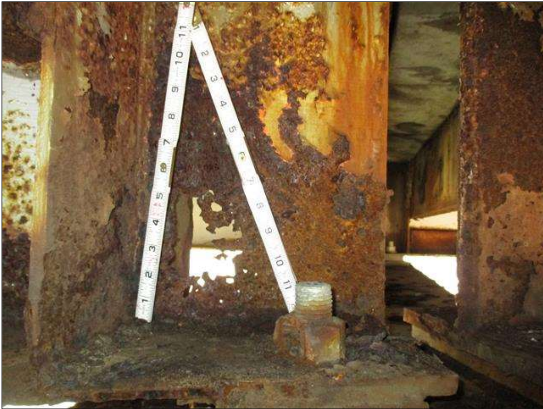
Span 2 Beam 3: (PAR) 100% SECTION LOSS FOR 7" LONG x 7" HIGH x 4" WIDE OVER BENT 2 BEARING
