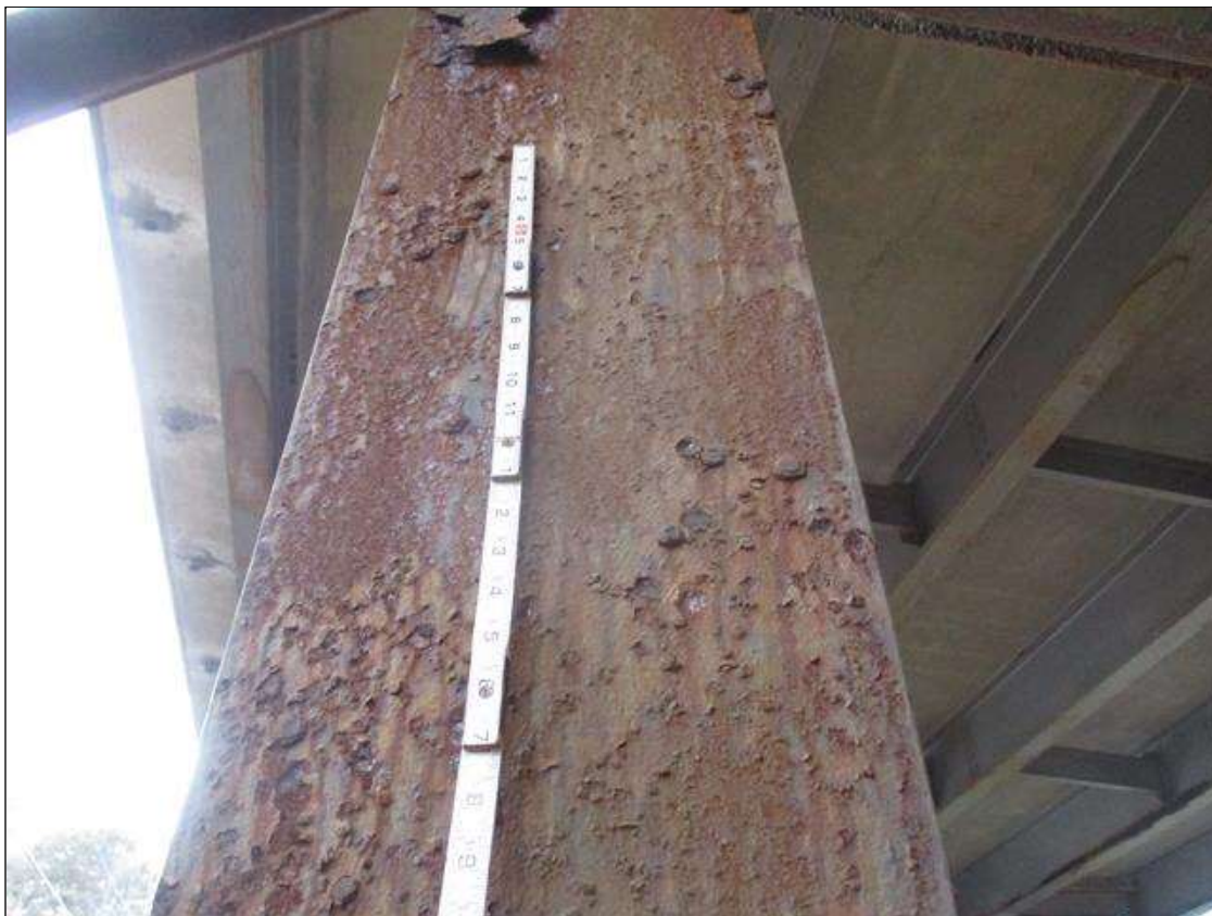
TYPICAL SURFACE CORROSION & DETERIORATED PAINT SYSTEM (BENT 3, PILE 9)
