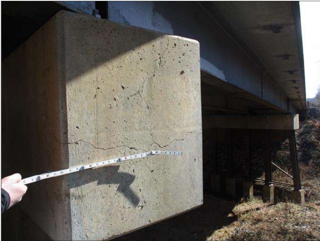
Bent 2 Cap 1: LONGITUDINAL CRACKING IN RIGHT END UP TO 1/16"
