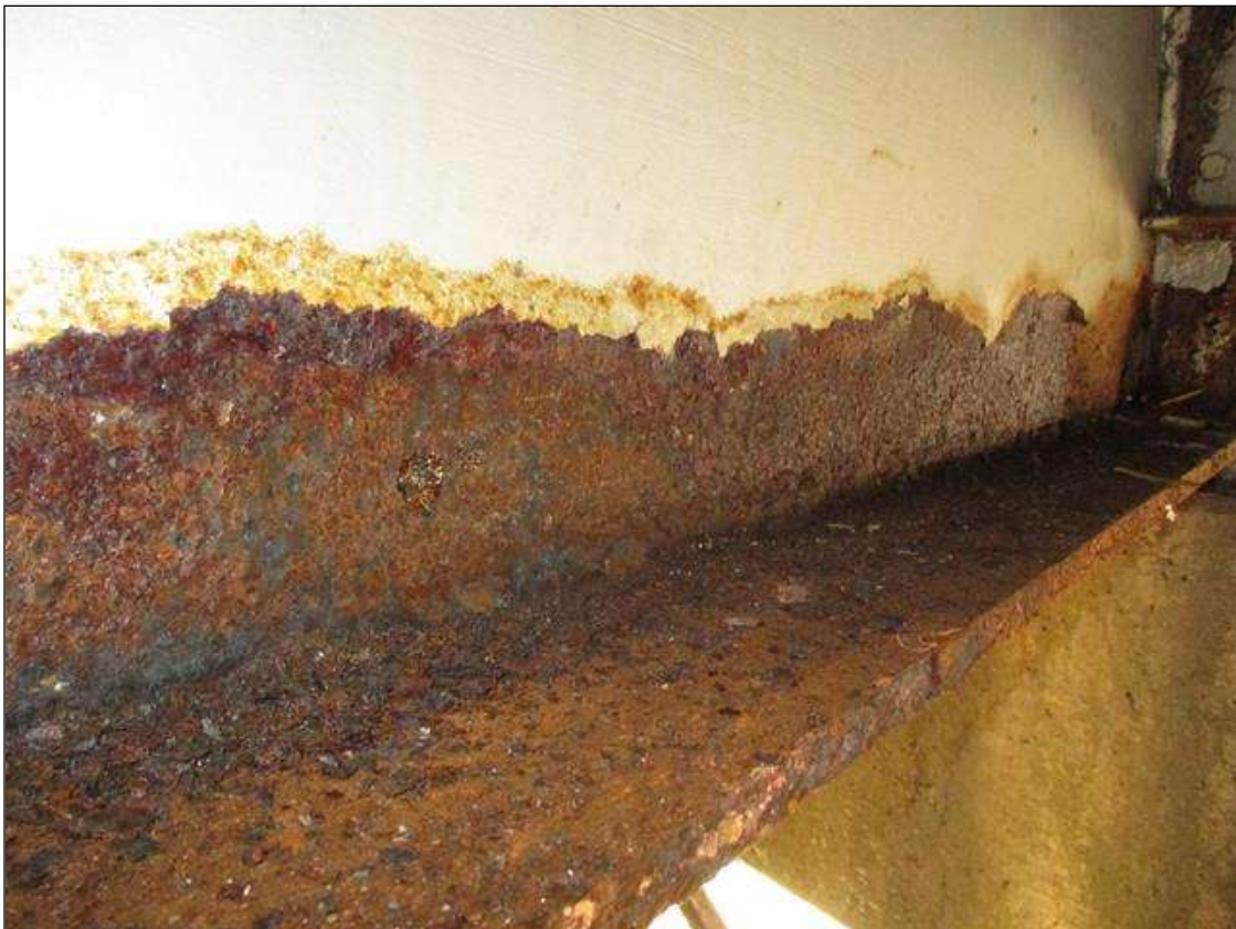
TYPICAL SURFACE CORROSION & DETERIORATED PAINT SYSTEM (SPAN 4, BEAM 2)
