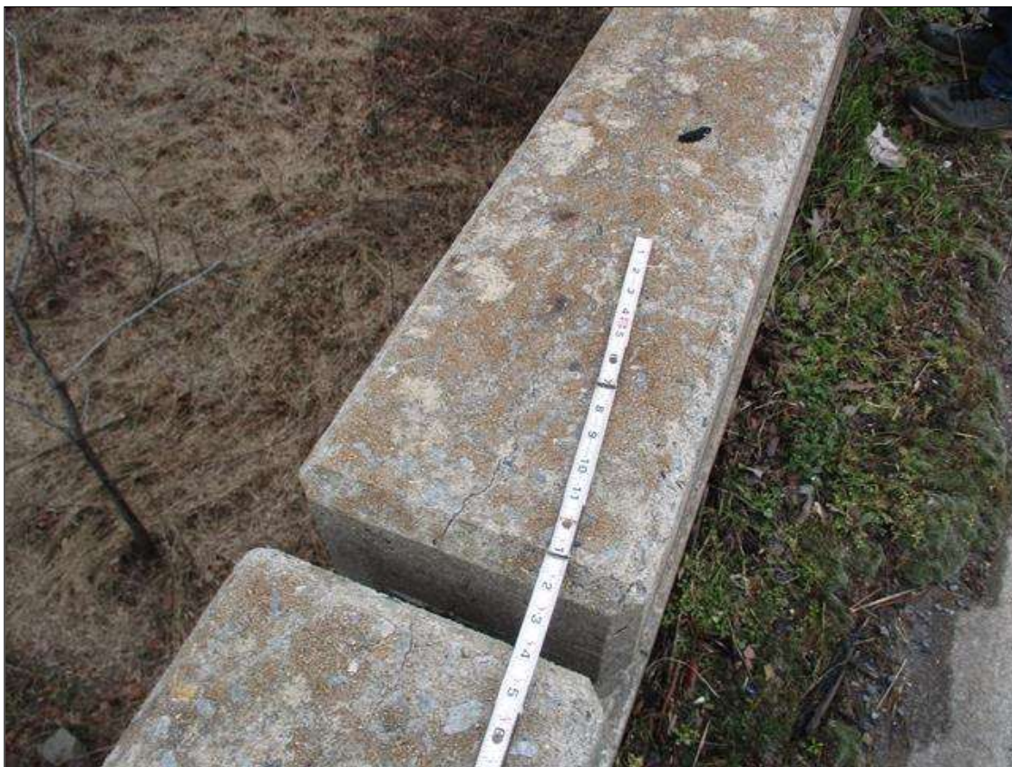
Span 4 Right Bridge Rail: UP TO 0.05" LONGITUDINAL AND VERTICAL CRACKS IN TOP AND ENDS OF RAIL IN VARIOUS LOCATIONS
