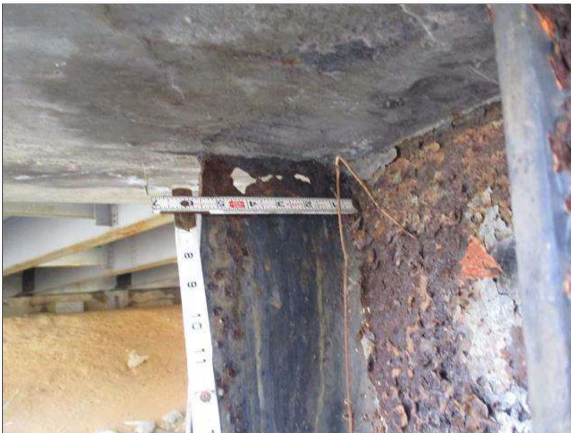
Bent 3 Pile 1: (PAR) CORROSION ALONG BOTH FLANGES UP TO 6" HIGH X 12" WIDE DOWN TO 3/8" RESIDUAL FLANGE AT BOTTOM OF CAP WITH UP TO 100% SECTION LOSS ON FAR FLANGE 4" WIDE X 1" HIGH ADJACENT TO CAP AND NEAR FLANGE
