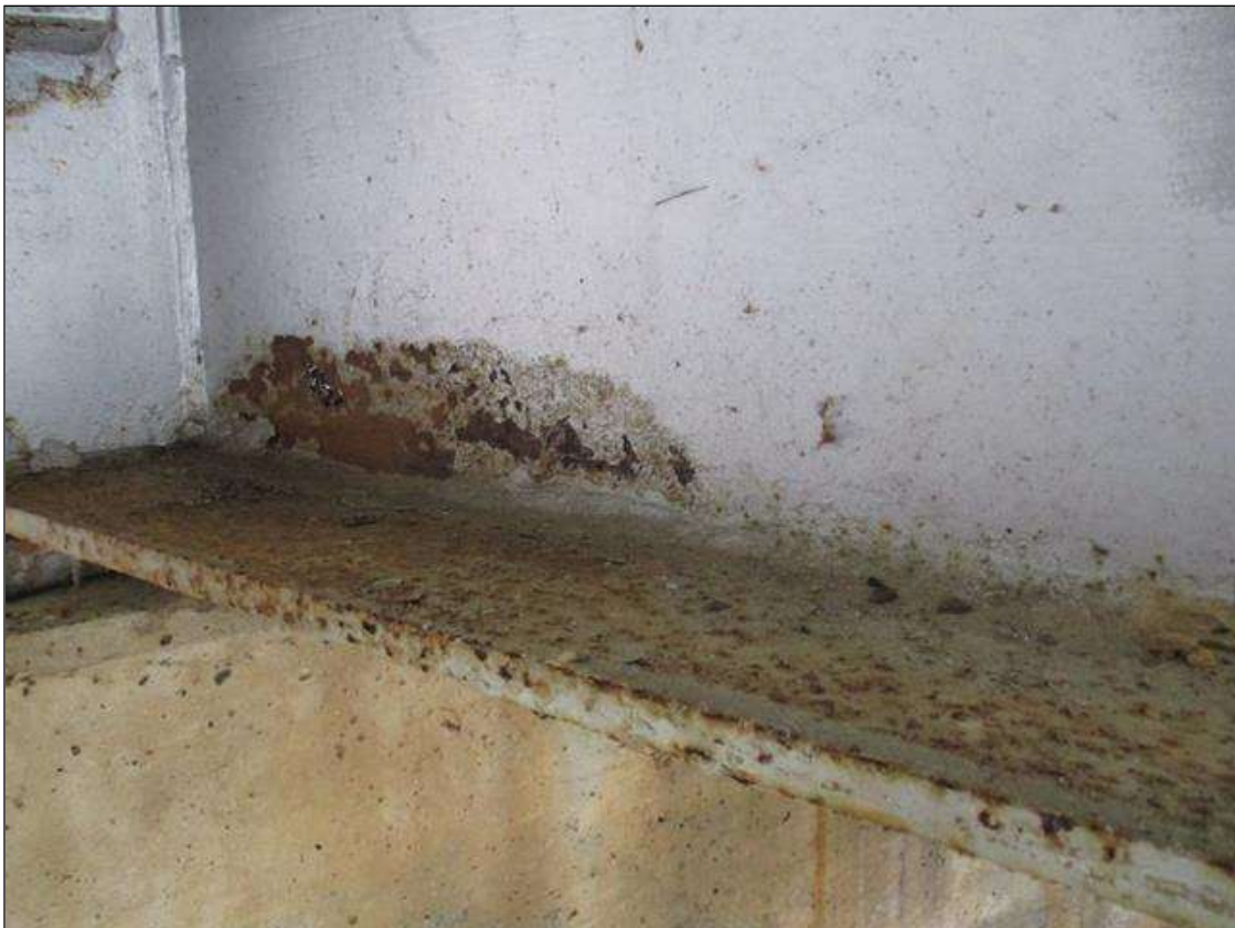
Span 2 Beam 4 - Protective System: DETERIORATED PAINT SYSTEM ALONG LEFT FACE OF WEB AND BOTTOM FLANGE UP TO 60" LONG X 5" HIGH IN WEB, AND 60" LONG X 11 3/4" WIDE IN FLANGE AT BENT 1 BEARING
