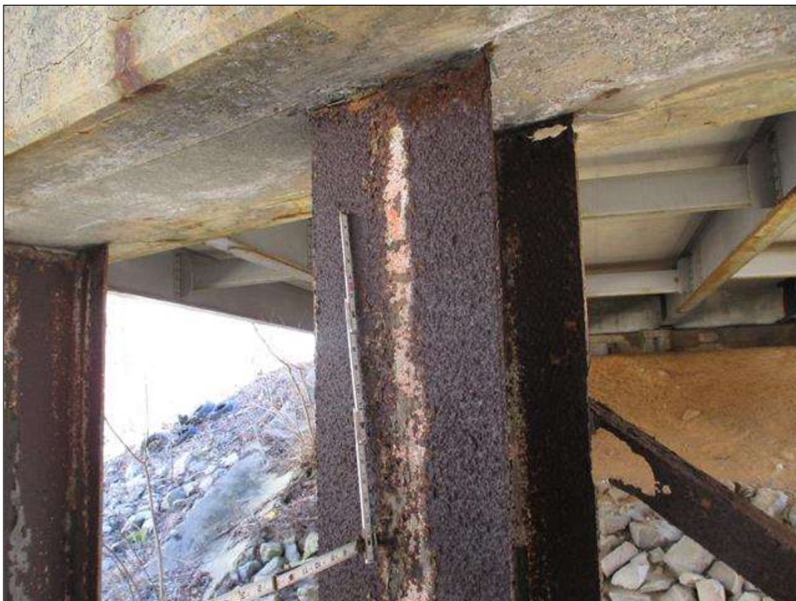
TYPICAL SURFACE CORROSION & DETERIORATED PAINT SYSTEM (BENT 3, PILE 5)
