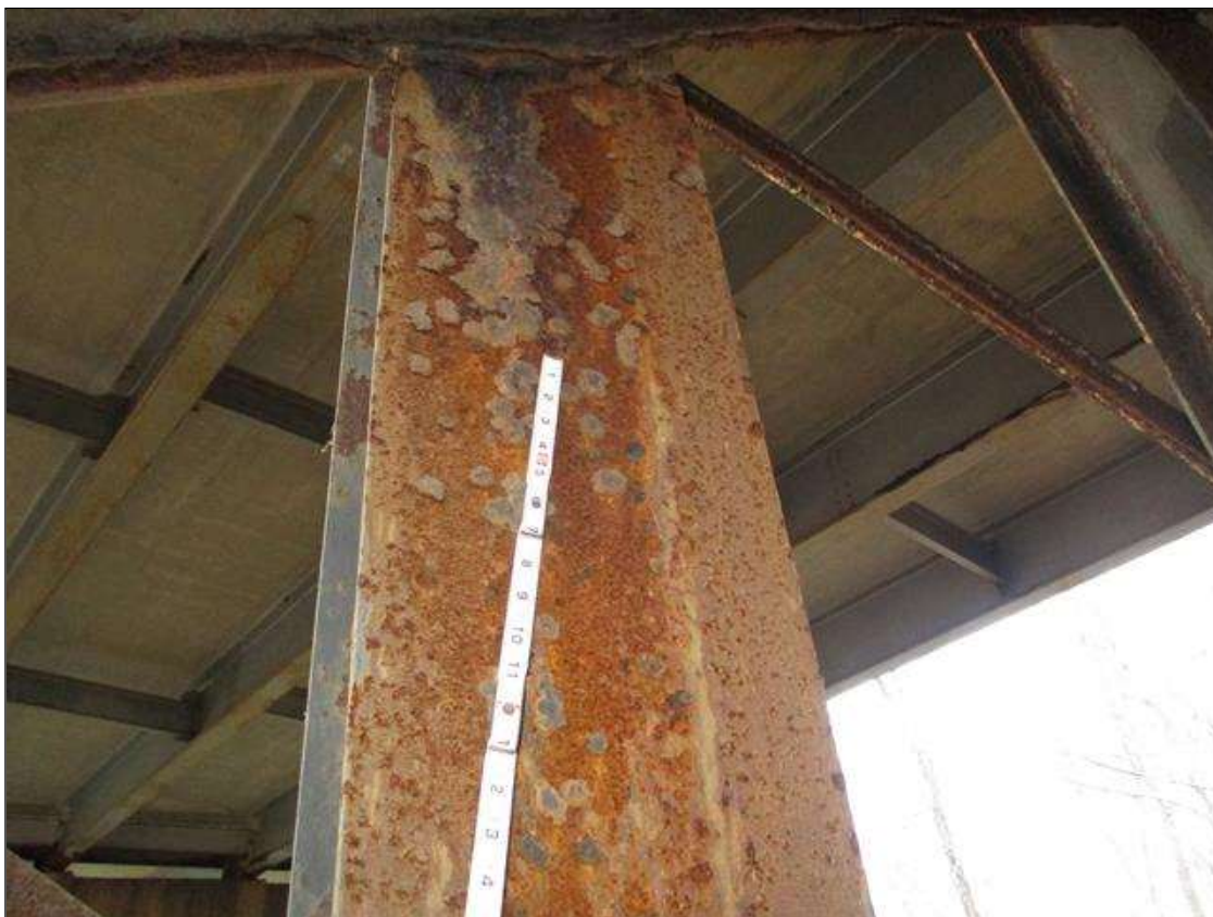
TYPICAL SURFACE CORROSION & DETERIORATED PAINT SYSTEM (BENT 3, PILE 7)
