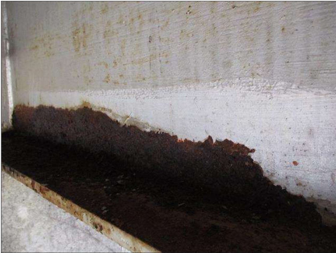
TYPICAL SURFACE CORROSION & DETERIORATED PAINT SYSTEM (SPAN 4, BEAM 1)
