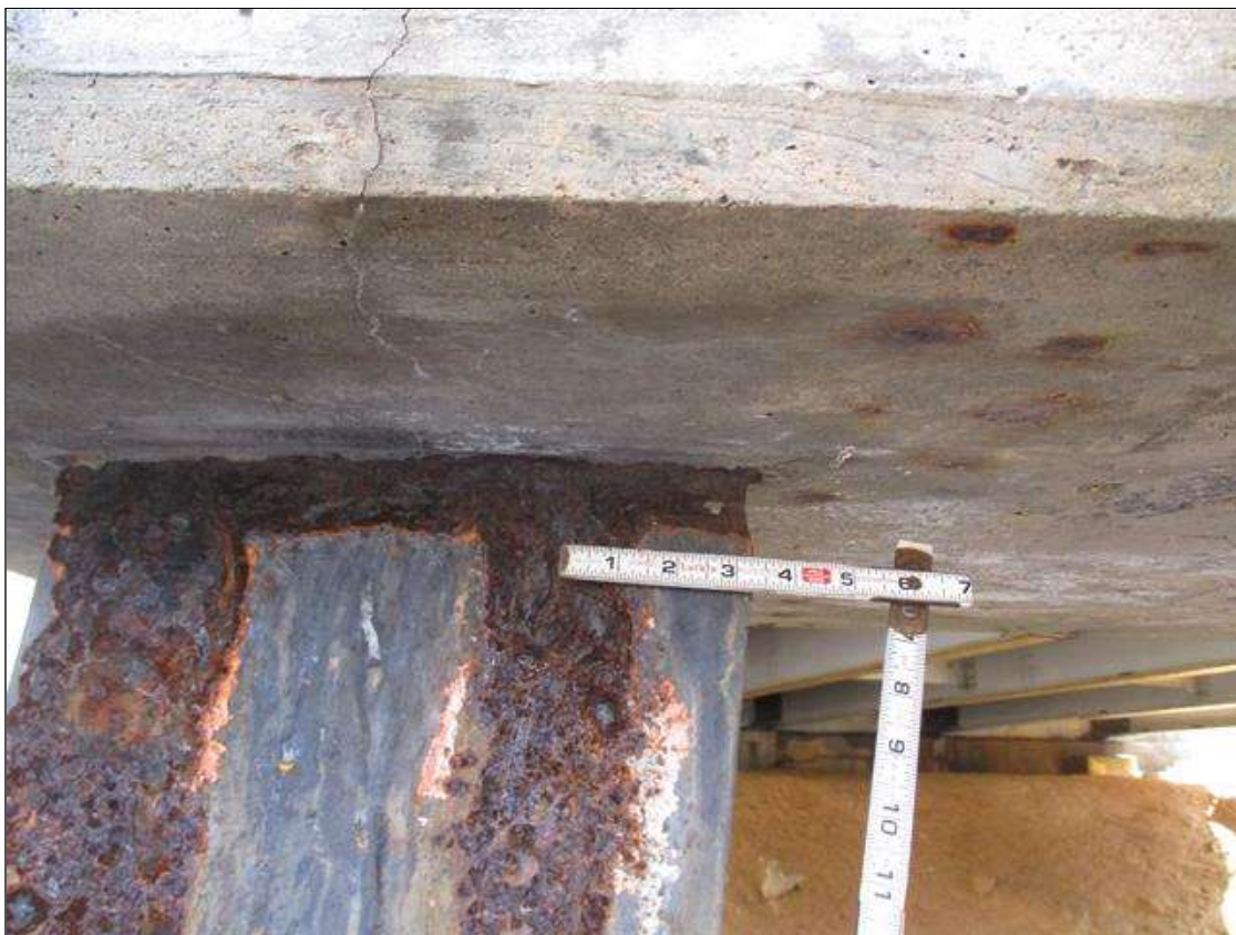
Bent 3 Pile 1: (PAR) CORROSION ALONG BOTH FLANGES UP TO 6" HIGH X 12" WIDE DOWN TO 3/8" RESIDUAL FLANGE AT BOTTOM OF CAP WITH UP TO 100% SECTION LOSS ON FAR FLANGE 4" WIDE X 1" HIGH ADJACENT TO CAP AND NEAR FLANGE
