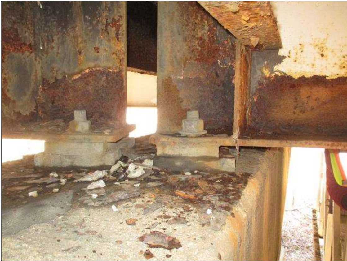
Span 4 Beam 4 - Near Bearing - Protective System: AREAS OF DETERIORATED PAINT SYSTEM THROUGHOUT BEAM 4 BEARING
