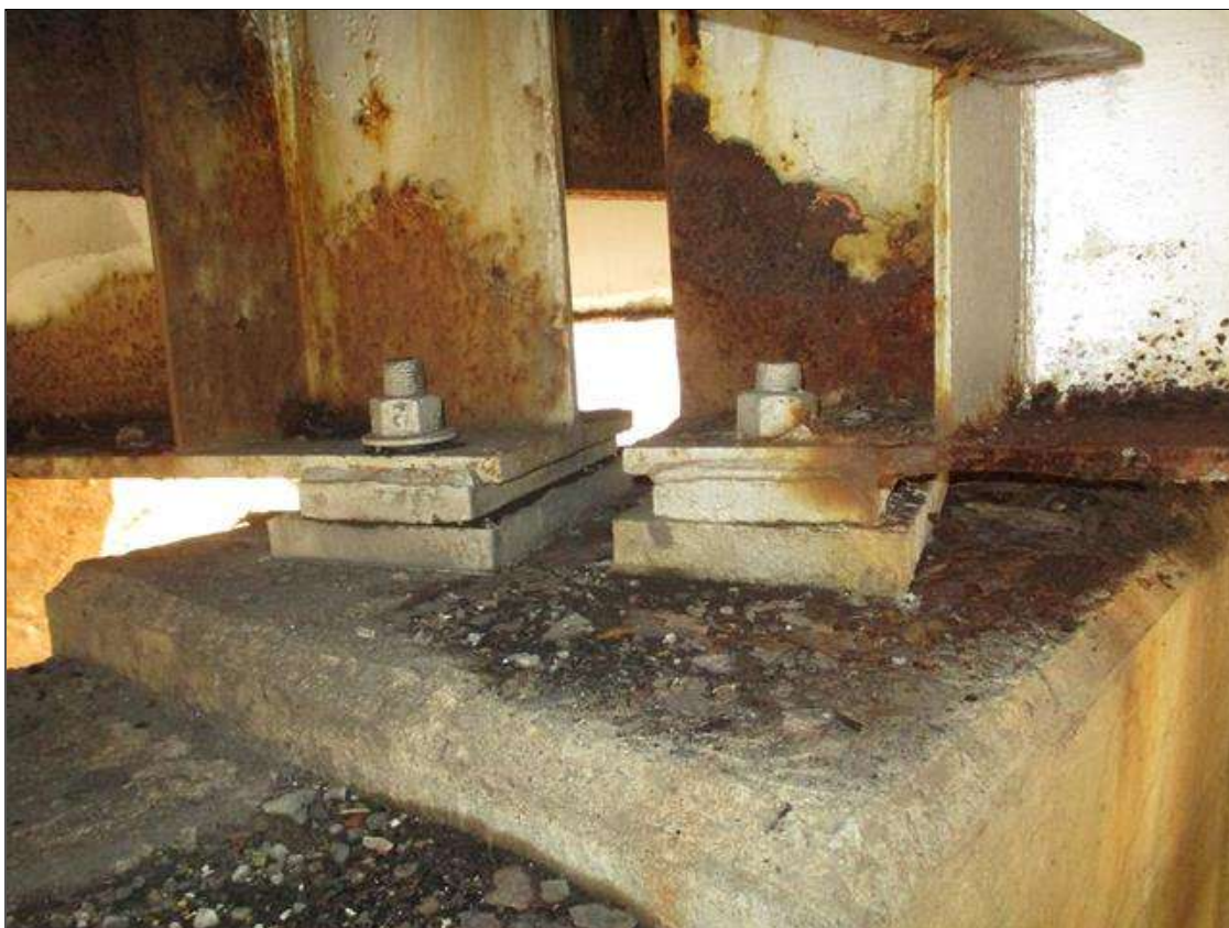
Span 3 Beam 1 - Far Bearing - Protective System: AREAS OF DETERIORATED PAINT SYSTEM THROUGHOUT BEAM 1 BEARING
