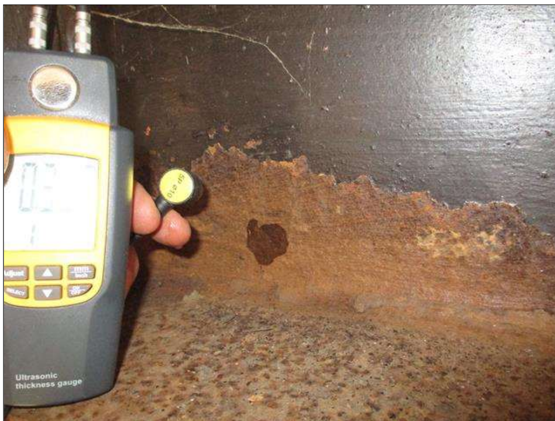
Span 3 Beam 6: (PAR) CORROSION ALONG BOTH FACES OF WEB AND BOTTOM FLANGE UP TO 20" LONG X 3" HIGH DOWN TO 0.362" RESIDUAL WEB, AND 11" LONG X 11 3/4" WIDE DOWN TO 0.543" RESIDUAL FLANGE AT BENT 3 BEARING
