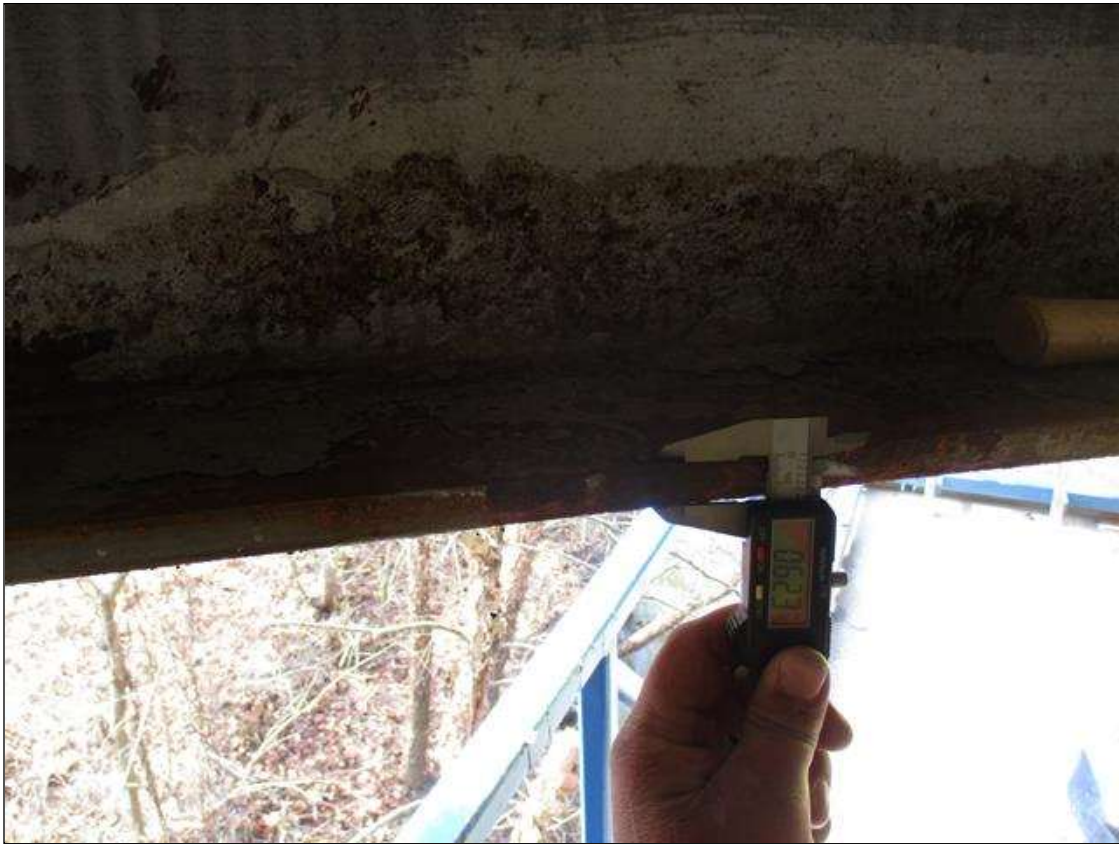
Span 3 Beam 6: 12' SECTION OF CORROSION ALONG LEFT FACE OF WEB AND BOTTOM FLANGE UP TO 4" HIGH WITH NO MEASURABLE LOSS OF SECTION IN WEB, AND 5" WIDE DOWN TO 0.623" RESIDUAL FLANGE, BEGINNING 7' FROM BENT 2 CAP
