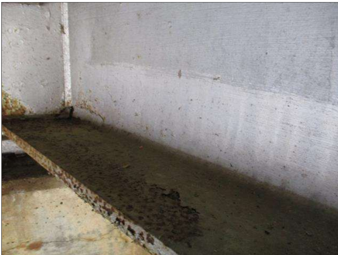
Span 2 Beam 4 - Protective System: AREAS OF DETERIORATED PAINT SYSTEM THROUGHOUT WEB AND BOTH FLANGES IN VARIOUS LOCATIONS
