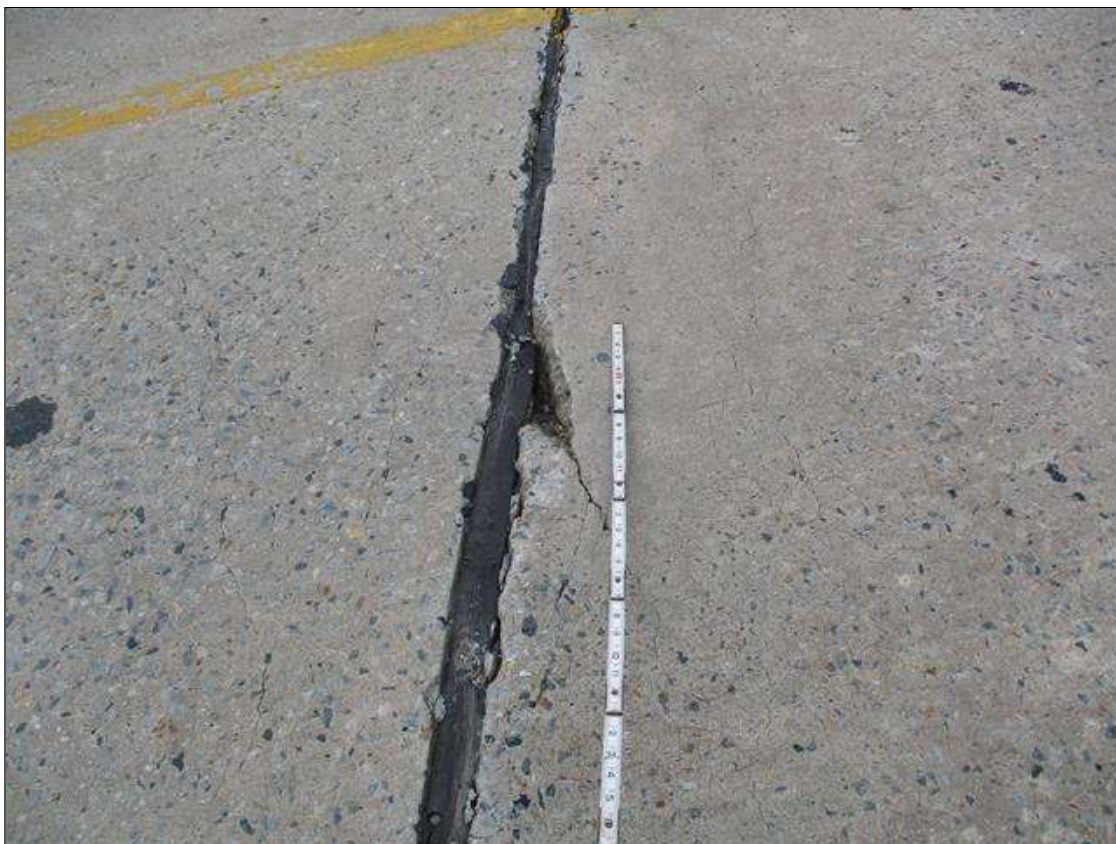
Span 1 Deck: AT BENT 1 JOINT, 10" X 3" X 3" DEEP SPALL IN TOP OF DECK IN WHEEL LINE OF WESTBOUND LANE
