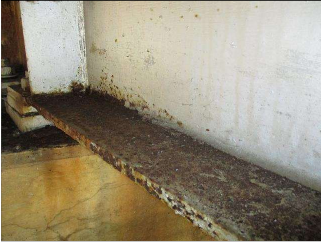
TYPICAL SURFACE CORROSION & DETERIORATED PAINT SYSTEM (SPAN 3, BEAM 2)
