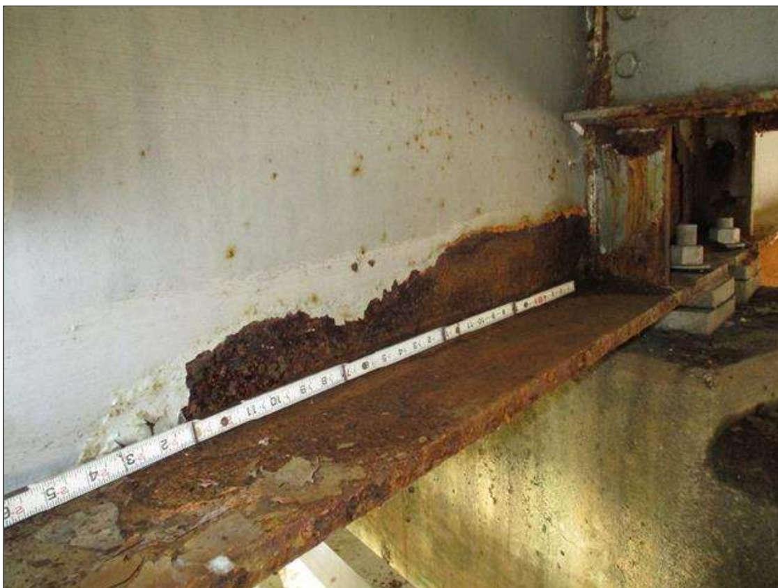
TYPICAL DETERIORATED PAINT SYSTEM (SPAN 2, BEAM 2)
