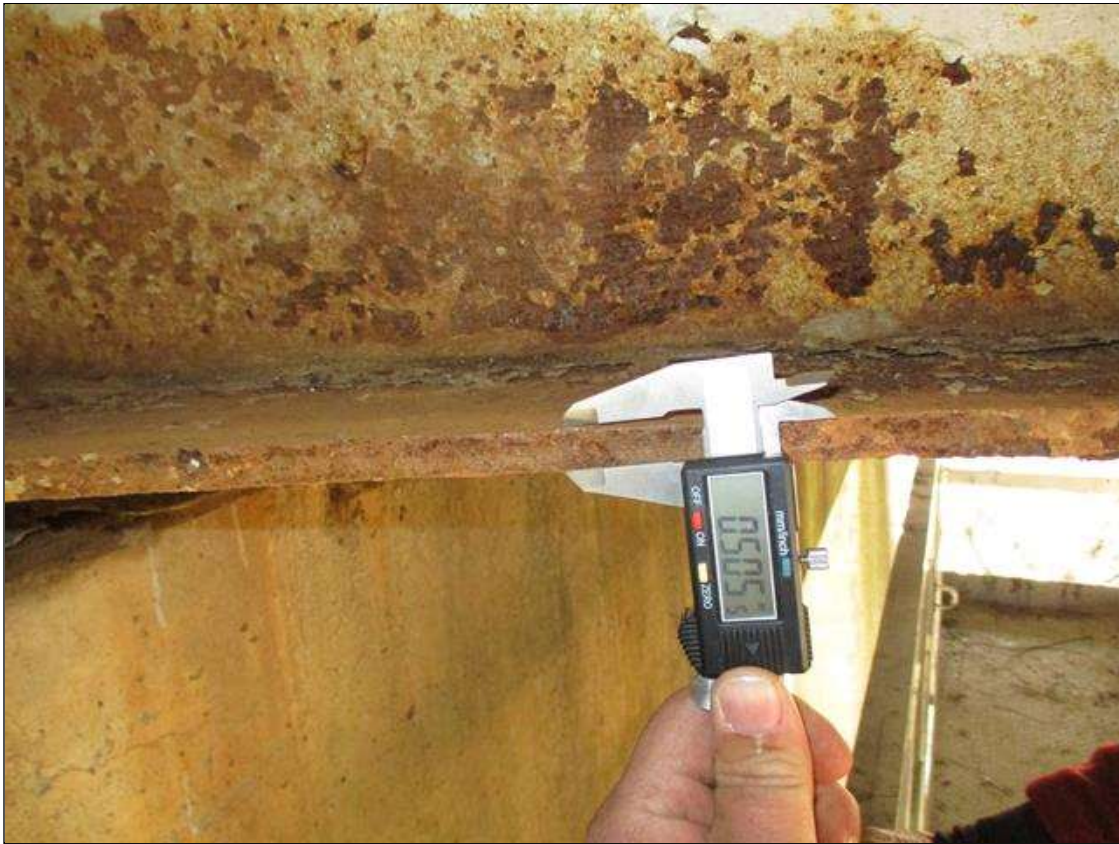
Span 3 Beam 4: (PAR) CORROSION ALONG BOTH FACES OF WEB AND BOTTOM FLANGE UP TO 58" LONG X 6" HIGH DOWN TO 0.342" RESIDUAL WEB, AND 39" LONG X 11 3/4" WIDE DOWN TO 0.505" RESIDUAL FLANGE AT BENT 2 BEARING
