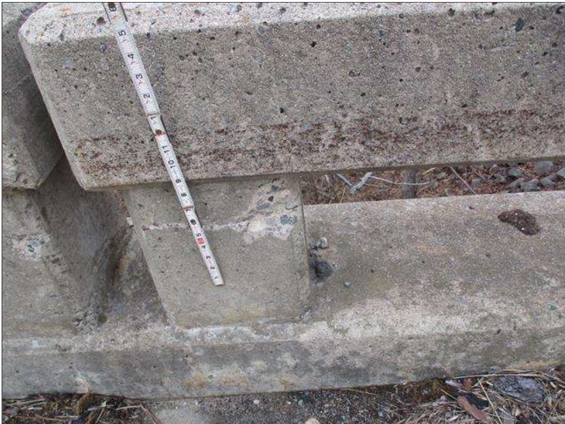
Span 4 Left Bridge Rail: FIVE (5) SPALLS UP TO 4" X 4" X 1/4" DEEP IN FACE OF RAIL POSTS IN VARIOUS LOCATIONS
