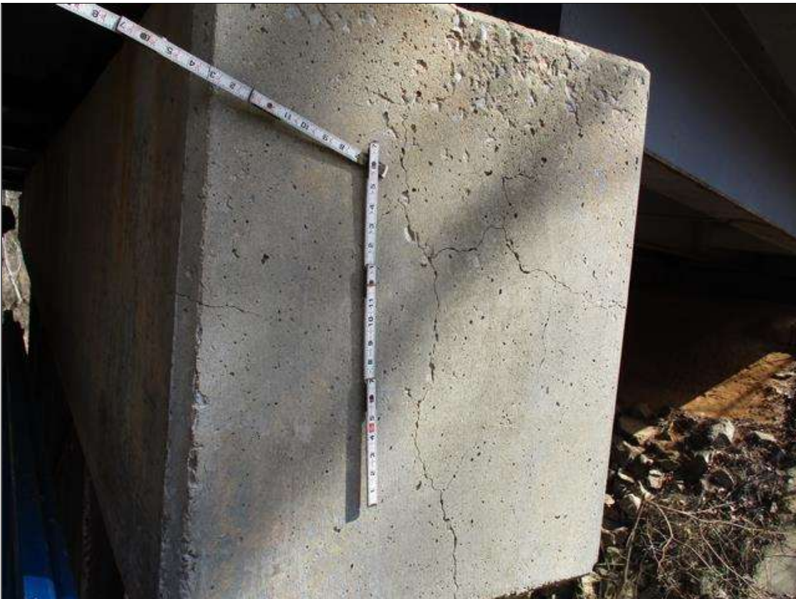
Bent 3 Cap 1: UP TO 1/4" LONGITUDINAL AND HORIZONTAL CRACKS AND HAIRLINE MAP CRACKING WITH AND WITHOUT EFFLORESCENCE IN BOTTOM AND BOTH FACES OF CAP
