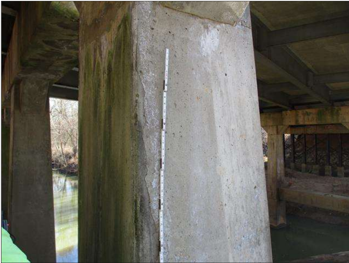
Bent 1 Pile 2: UP TO 48" X 1/8" VERTICAL CRACKS THROUGHOUT COLUMN AT WATER SURFACE
