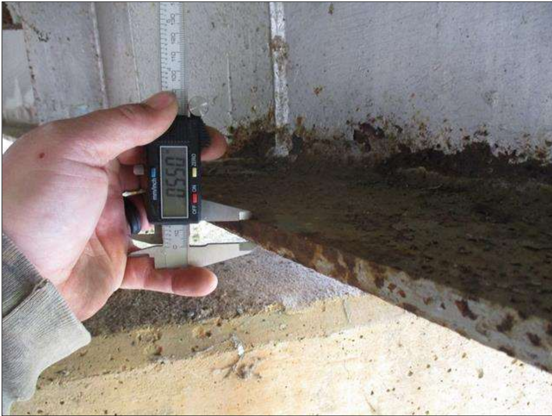
Span 2 Beam 6: CORROSION ALONG LEFT FACE OF WEB AND BOTTOM FLANGE UP TO 22" LONG X 4" HIGH WITH NO MEASURABLE LOSS OF SECTION IN WEB, AND 14" LONG X 5" WIDE DOWN TO 0.550" RESIDUAL FLANGE AT BENT 2 BEARING
