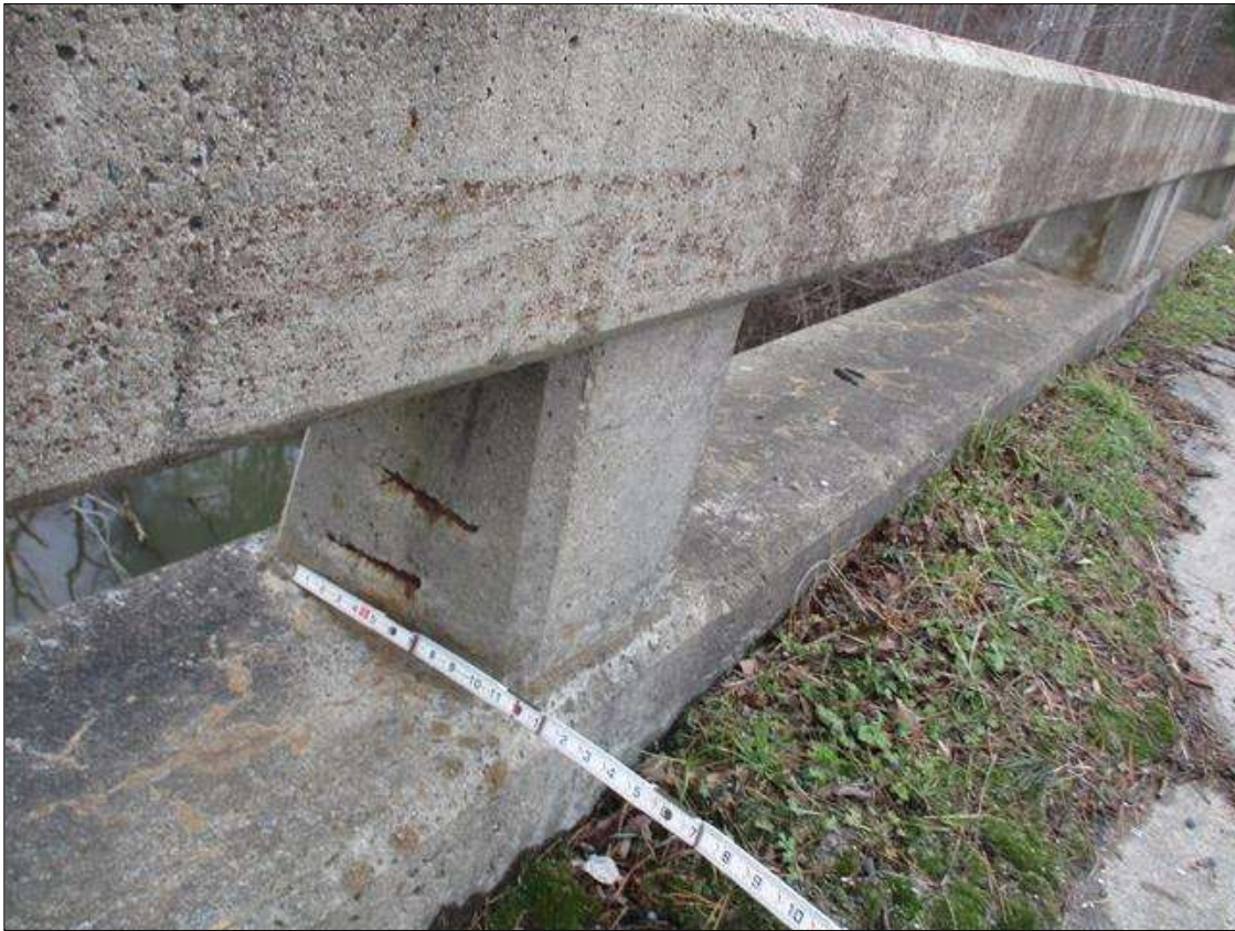
Span 2 Right Bridge Rail: TWO (2) SPALLS WITH EXPOSED REBAR UP TO 5" X 1 1/2" X 1/4" DEEP IN EAST FACE OF RAIL POST NEAR MIDSPAN
