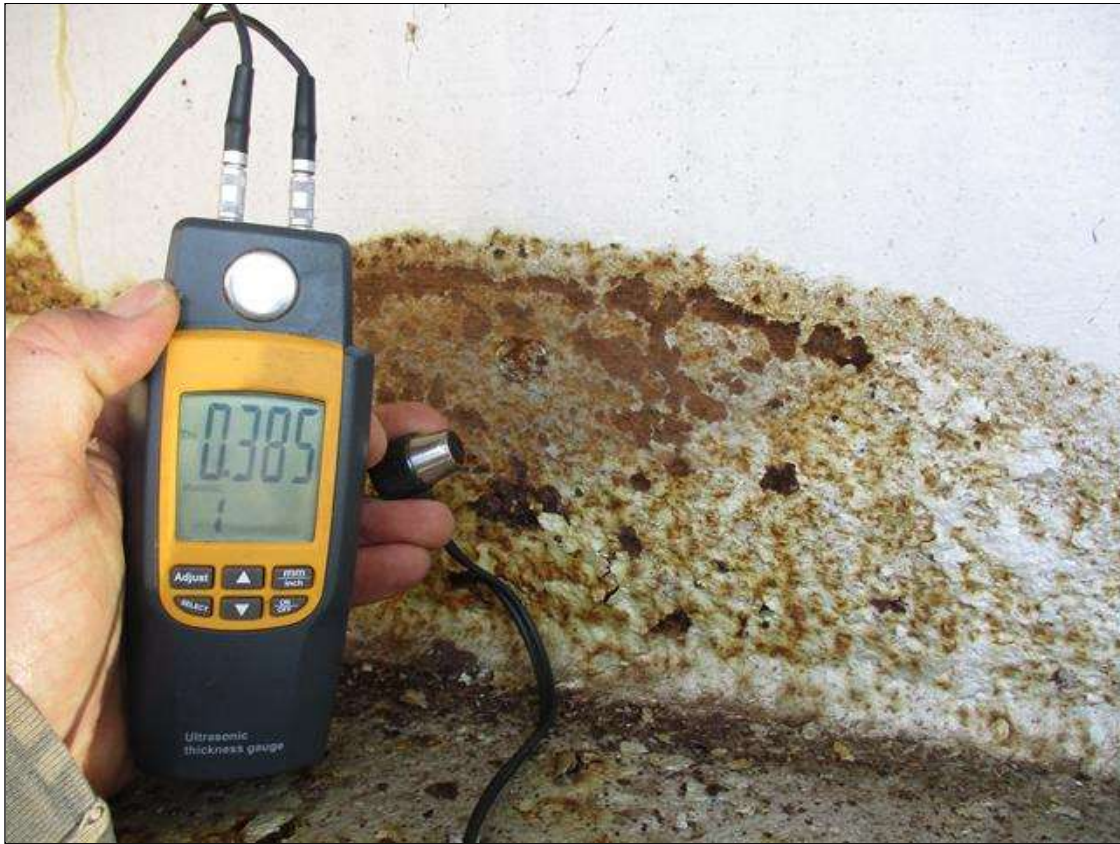
Span 2 Beam 6: (PAR) CORROSION ALONG BOTH FACES OF WEB AND BOTTOM FLANGE UP TO 58" LONG X 7" HIGH DOWN TO 0.385" RESIDUAL WEB, AND 67" LONG X 11 1/2" WIDE DOWN TO 9/16" RESIDUAL FLANGE AT BENT 1 BEARING
