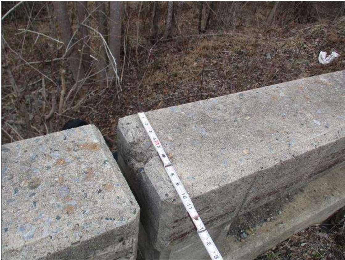
Span 4 Left Bridge Rail: 4" X 1 1/2" X 2" SPALL IN TOP AND WEST END OF RAIL, APPROXIMATELY 17' FROM END BENT 2 FILL FACE
