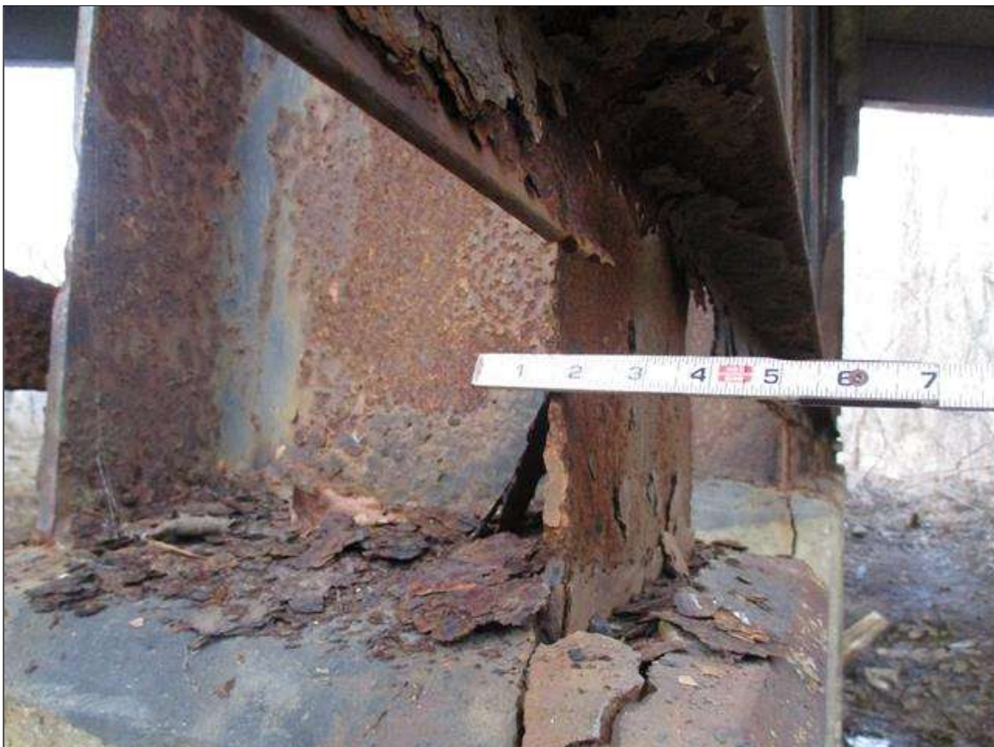
Bent 3 Pile 8: (PAR) CORROSION ALONG BOTH FLANGES UP TO 20" HIGH X 12" WIDE DOWN TO KNIFE'S EDGE RESIDUAL FLANGE ABOVE CONCRETE ENCASEMENT
