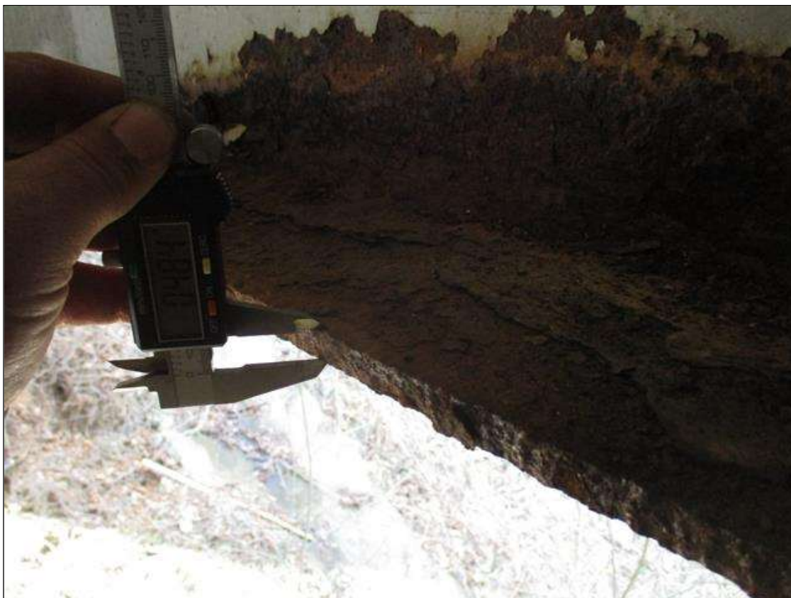
Span 1 Beam 2: (PAR) CORROSION ALONG RIGHT FACE OF WEB AND BOTTOM FLANGE UP TO 39" LONG X 10" HIGH DOWN TO 0.3" RESIDUAL WEB, AND 35" LONG X 5" WIDE DOWN TO 0.48" RESIDUAL FLANGE AT BENT 1 BEARING
