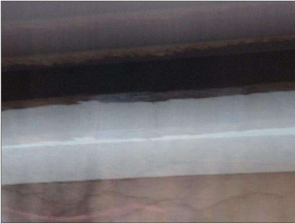
(PAR) STEEL DIAPHRAGM: SPAN 2 AT BENT 1 IN BAY 3, CORROSION ALONG TOP FLANGE UP TO 36" LONG X 1" WIDE WITH NO MEASURABLE LOSS OF SECTION, AND CORROSION ALONG BOTTOM FLANGE UP TO 22" X 3" DOWN TO KNIFE'S EDGE RESIDUAL FLANGE WITH 4" LONG X 1" WIDE LOSS OF SECTION NEAR MIDLNGTH
