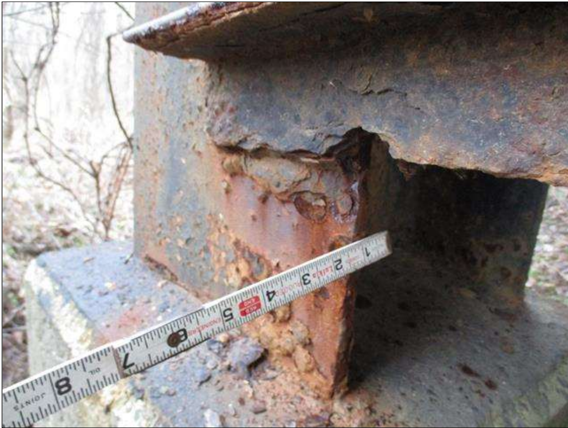
Bent 3 Pile 1: (PAR) CORROSION ALONG RIGHT EDGE OF NEAR FLANGE UP TO 23" HIGH X 6" WIDE DOWN TO 3/8" RESIDUAL FLANGE ABOVE CONCRETE ENCASEMENT
