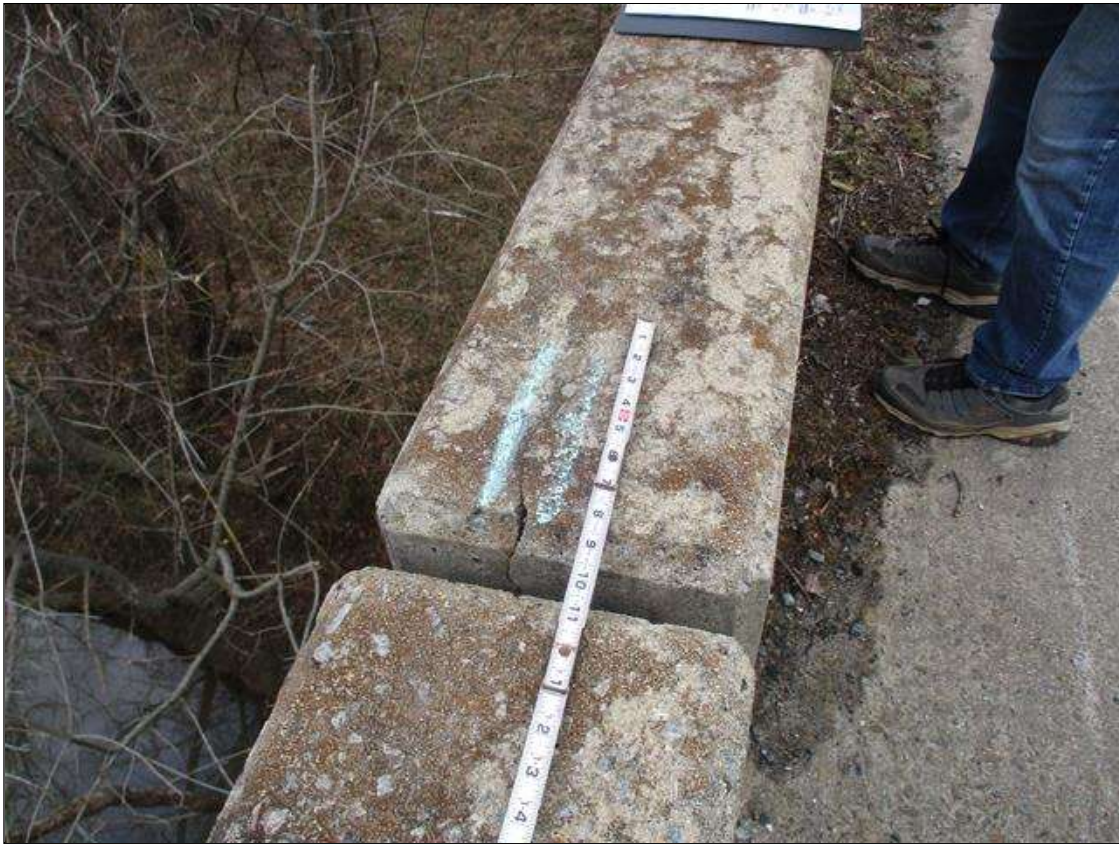
Span 3 Left Bridge Rail: UP TO 0.035" LONGITUDINAL AND VERTICAL CRACKS IN TOP AND ENDS OF RAIL IN VARIOUS LOCATIONS
