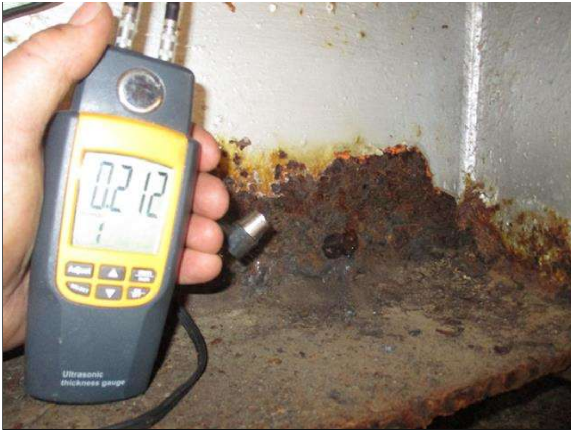
Span 3 Beam 2: (PAR) CORROSION ALONG BOTH FACES OF WEB AND BOTTOM FLANGE UP TO 32" LONG X 5" HIGH DOWN TO 0.212" RESIDUAL WEB, AND 34" LONG X 11 3/4" WIDE DOWN TO 0.350" RESIDUAL FLANGE AT BENT 3 BEARING
