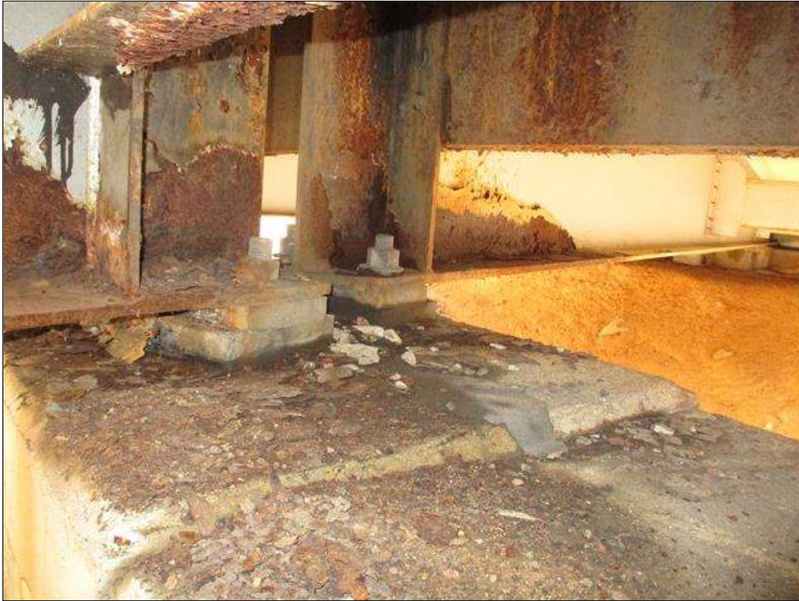
Span 3 Beam 5 - Far Bearing - Protective System: AREAS OF DETERIORATED PAINT SYSTEM THROUGHOUT BEAM 5 BEARING
