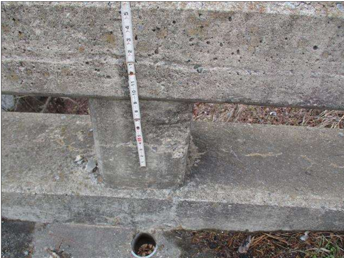
Span 1 Right Bridge Rail: 4" X 2" X 1/2" DEEP SPALL WITH EXPOSED REBAR IN EAST OF RAIL POST, APPROXIMATELY 9' FROM END BENT 1 FILL FACE
