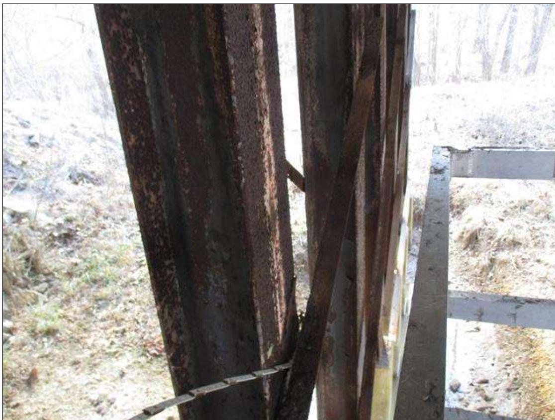
(PAR) AREAS OF 100% SECTION LOSS UP 17" X 3" AND BROKEN AND DETACHED CROSS BRACING INTERMITTENT THROUGHOUT BENT 3
