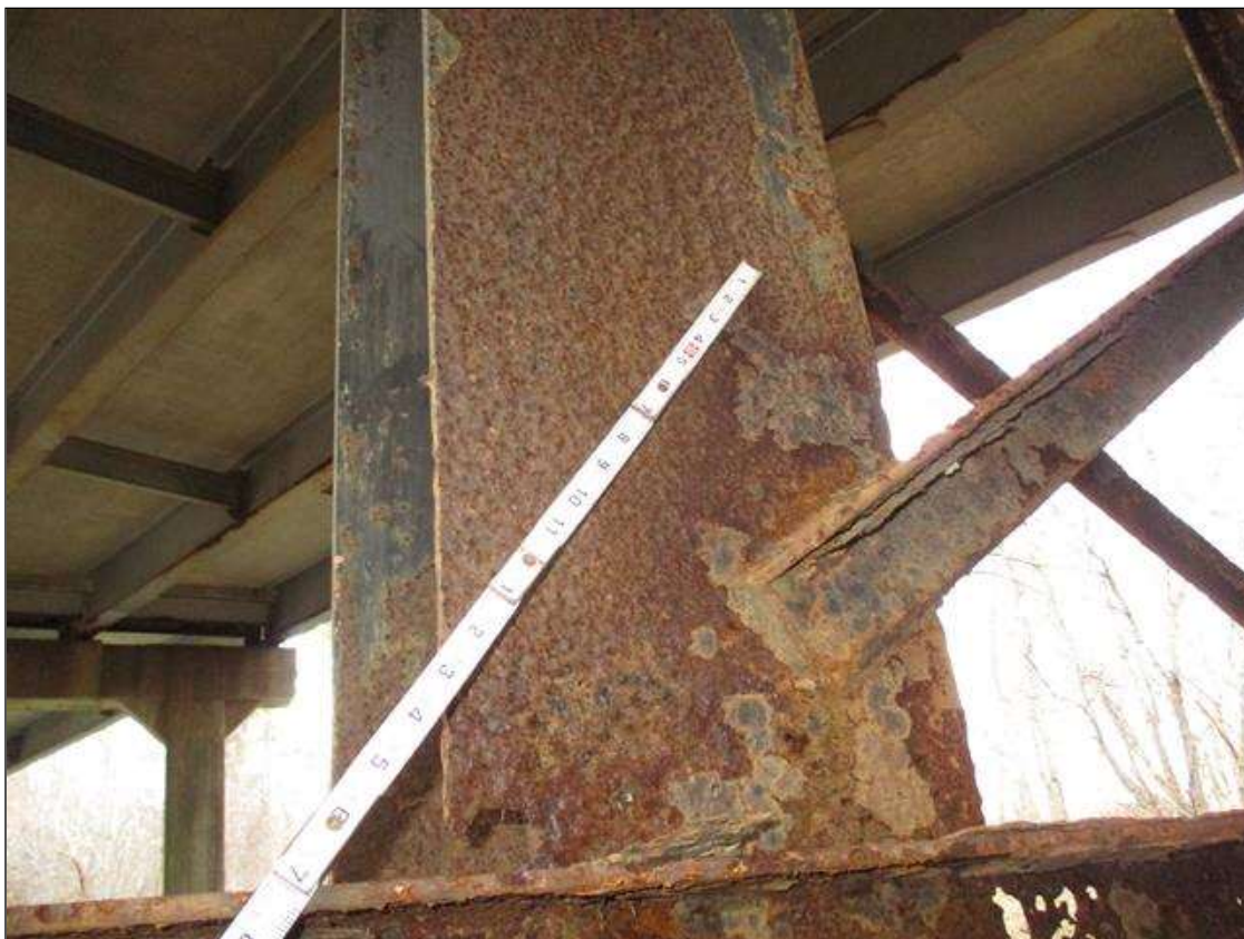
TYPICAL SURFACE CORROSION & DETERIORATED PAINT SYSTEM (BENT 3, PILE 6)
