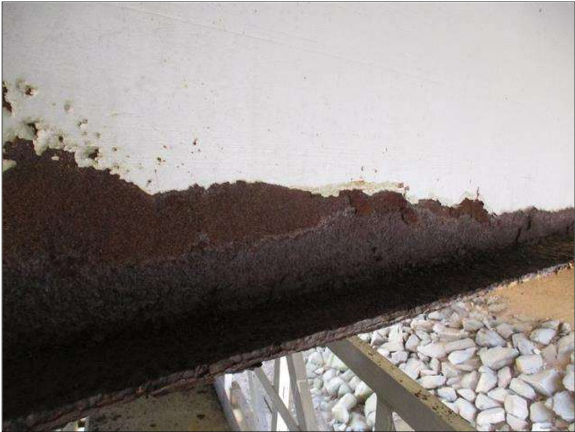
TYPICAL SURFACE CORROSION & DETERIORATED PAINT SYSTEM (SPAN 4, BEAM 5)
