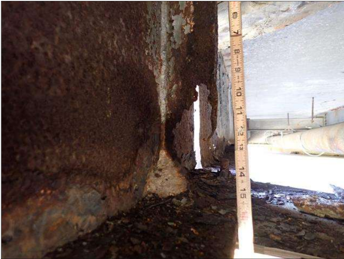
Span 2 Beam 7: PAR: CORROSION THROUGHOUT LEFT SIDE STIFFENER WITH 7 INCH X 4 INCH LOSS OF SECTION AT BENT 1 BEARING
