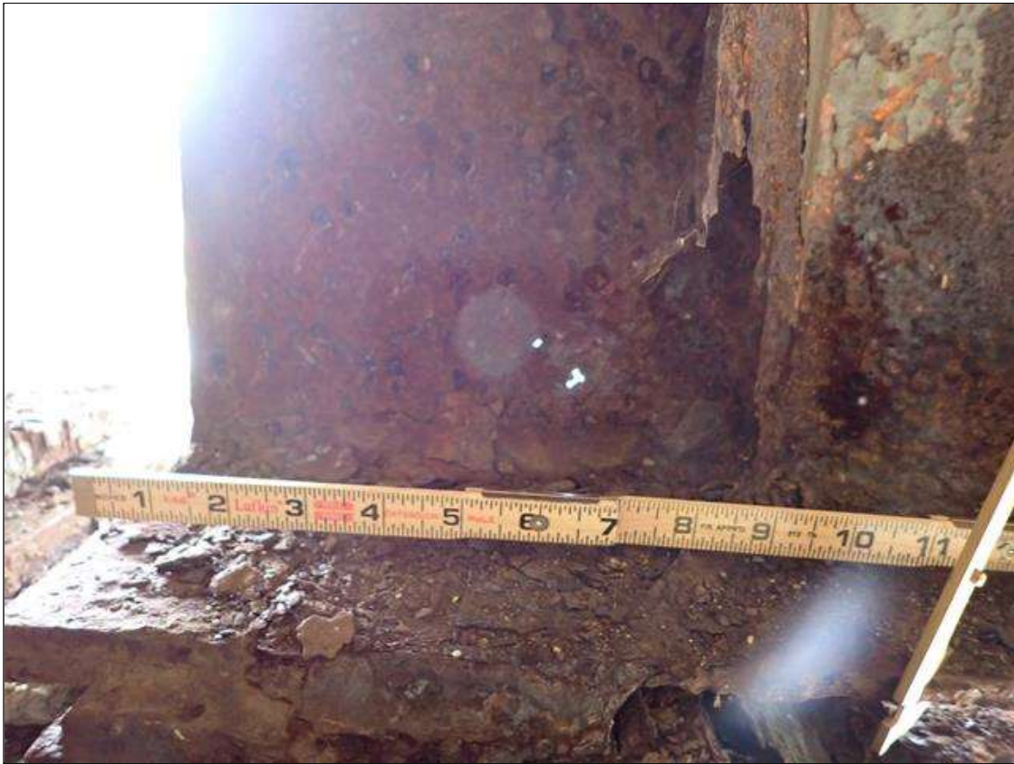
Span 4 Beam 1: PAR: CORROSION ALONG BOTH FACES OF WEB AND BOTTOM FLANGE UP TO 68 INCH LONG X UP TO 20 INCH HIGH DOWN TO 1/4 INCH RESIDUAL WEB WITH PIN HOLES BEHIND STIFFENER AND 52 INCH LONG X 10 INCH WIDE DOWN TO 5/16 INCH RESIDUAL BOTTOM FLANGE EXTENDING FROM BENT 3
