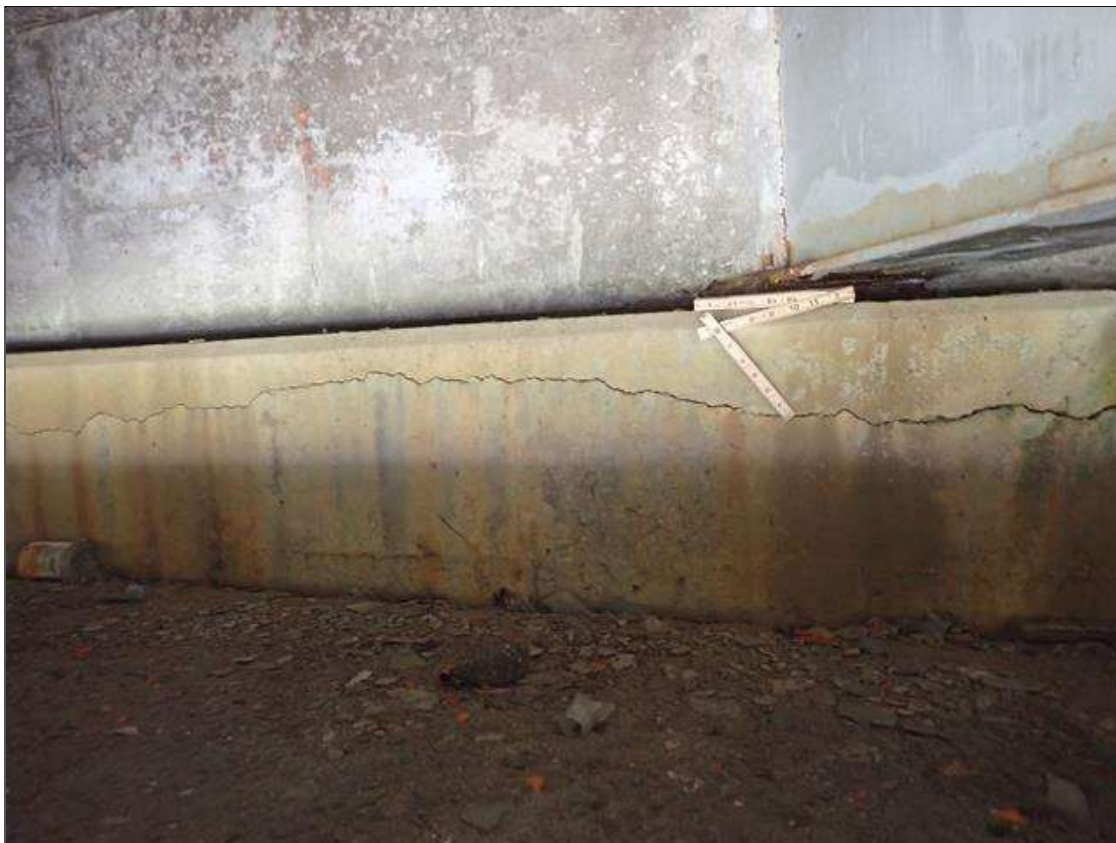
End Bent 1 Cap 1: UP TO 1/8 INCH X 15 FOOT LONG HORIZONTAL CRACK IN FACE OF CAP BENEATH BEAMS 3 AND 4
