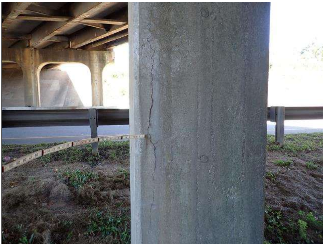
Bent 2 Pile 3: UP TO 1/16 INCH VERTICAL CRACK IN SPAN 2 FACE ALONG LEFT EDGE AT MID HEIGHT
