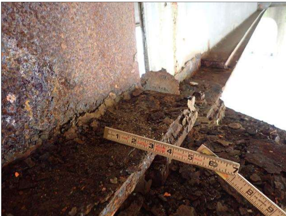
Span 4 Beam 4 - Near Bearing: PAR: MISSING ANCHOR ROD ON WEST SIDE
