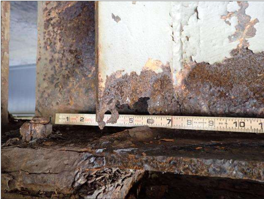
Span 2 Beam 5: PAR: CORROSION THROUGHOUT RIGHT SIDE STIFFENER WITH 4 INCH X 2 INCH LOSS OF SECTION AT BENT 1 BEARING
