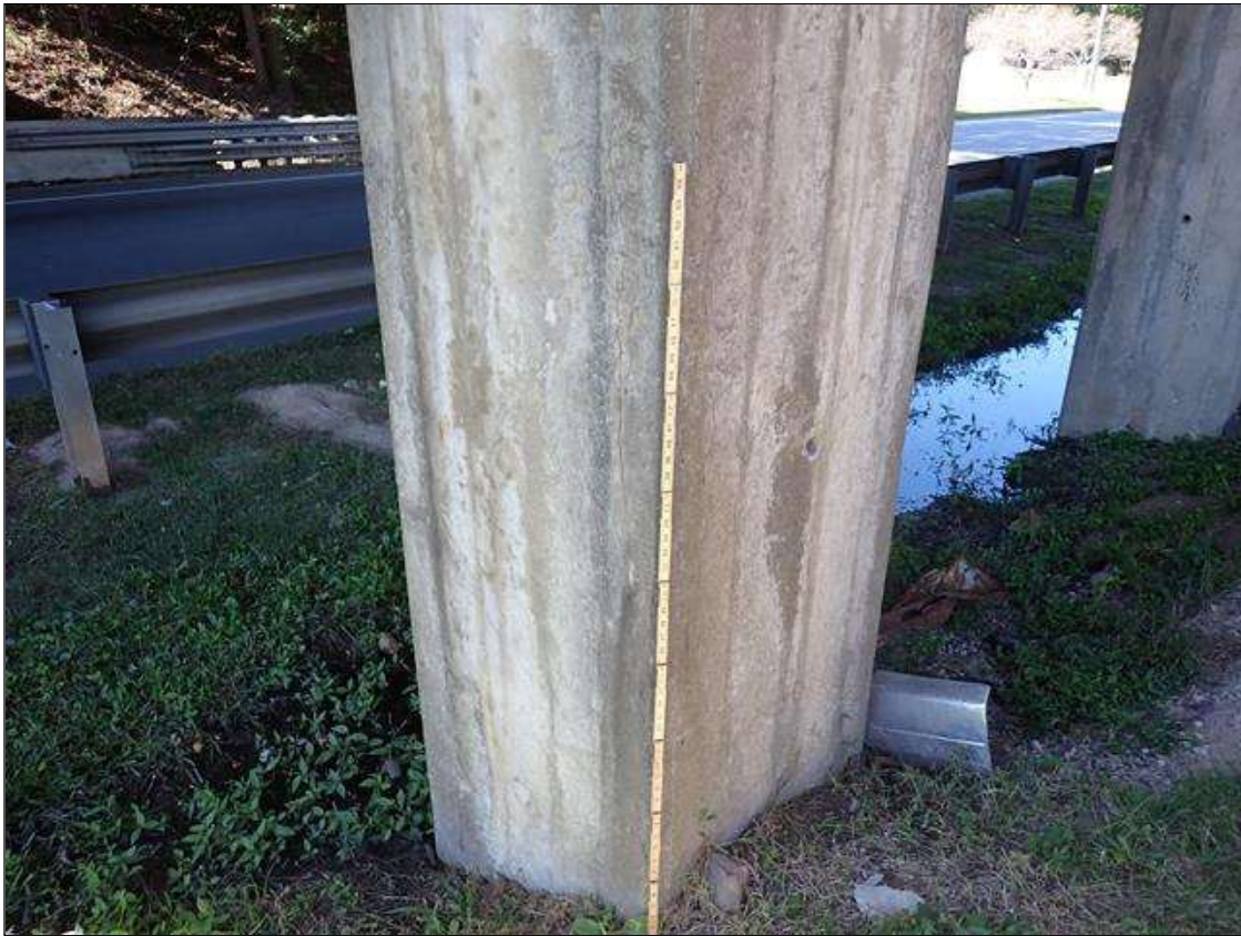
Bent 2 Pile 5: UP TO 1/16 INCH X 40 INCH VERTICAL CRACKS IN SPAN 3 AND EAST FACE OF COLUMN NEAR GROUND LINE
