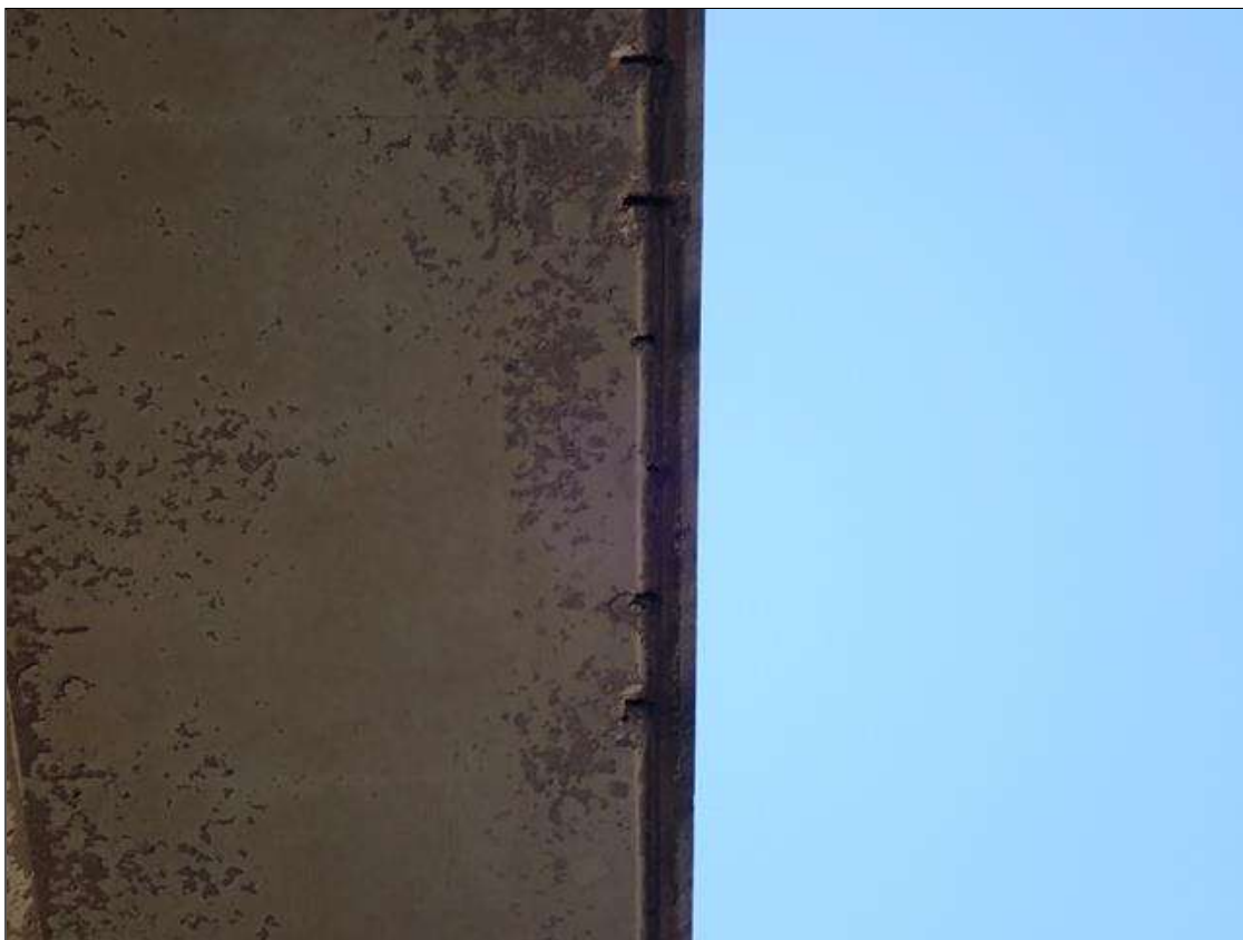
Span 2 Deck: (20) 4 INCH X 1 INCH X 1/2 INCH SPALLS WITH EXPOSED REINFORCING, AT RANDOM ALONG EAST EDGE OF EAST OVERHANG
