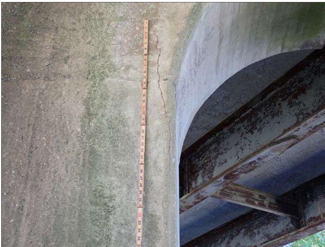
Bent 2 Pile 3: UP TO 1/16 INCH X 28 INCH VERTICAL CRACK IN NORTHWEST CORNER AT BOTTOM OF CAP
