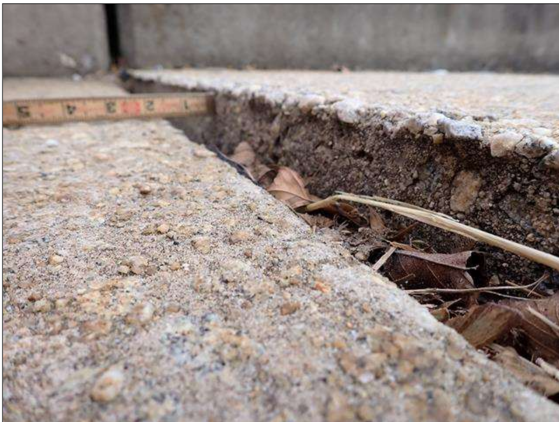
SAG ALONG RIGHT SIDE OF SPAN 3 DECK AND RAIL ABOVE BEAM 7 WITH VERTICAL DEFLECTION OF DECK AND SIEWALK AT BENT 3
