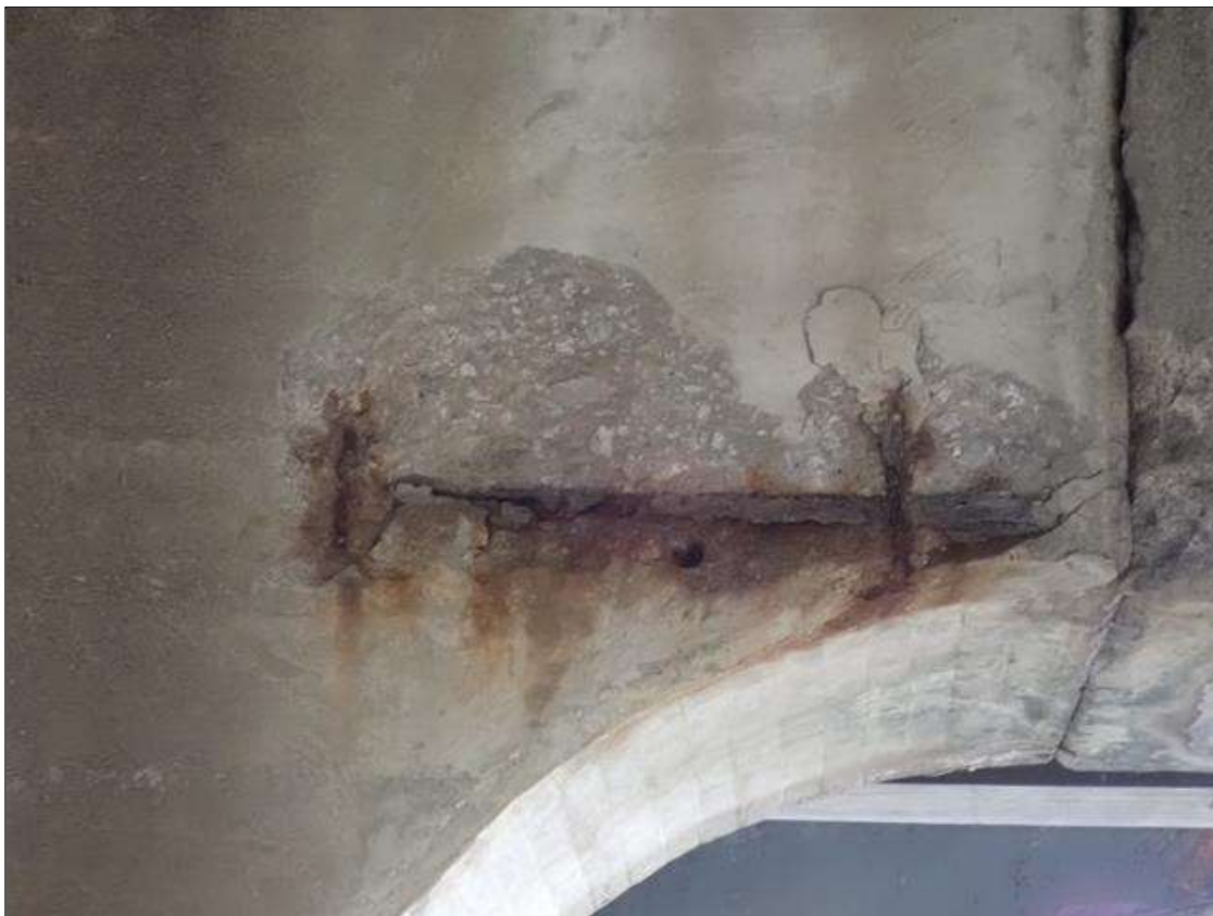
Bent 3 Cap 1: PAR: 28 INCH LONG X 12 INCH HIGH X 2 INCH DEEP SPALL WITH EXPOSED REBAR IN SPAN 4 FACE OF CAP BENEATH BEAM 3
