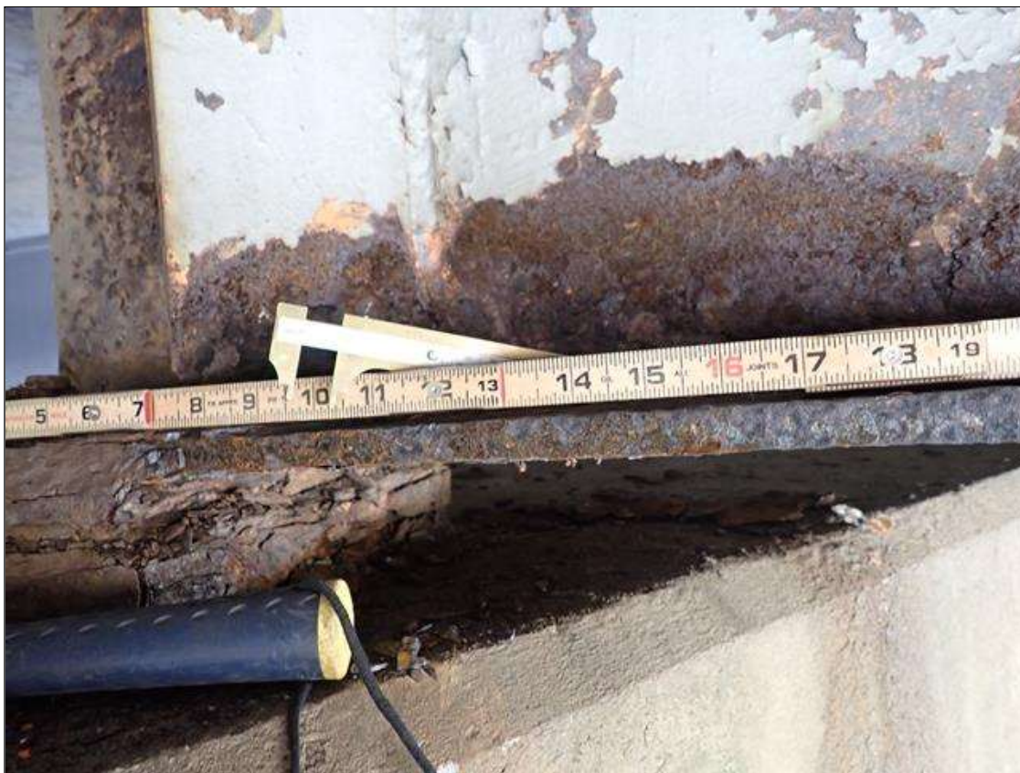
Span 2 Beam 5: PAR: CORROSION ALONG BOTH FACES OF WEB AND BOTTOM FLANGE UP TO 36 INCH LONG X UP TO 17 INCH HIGH WITH NO MEASURABLE LOSS OF SECTION IN RESIDUAL WEB AND 18 INCH LONG X 10 INCH WIDE DOWN TO 9/16 INCH RESIDUAL BOTTOM FLANGE EXTENDING FROM BENT 1
