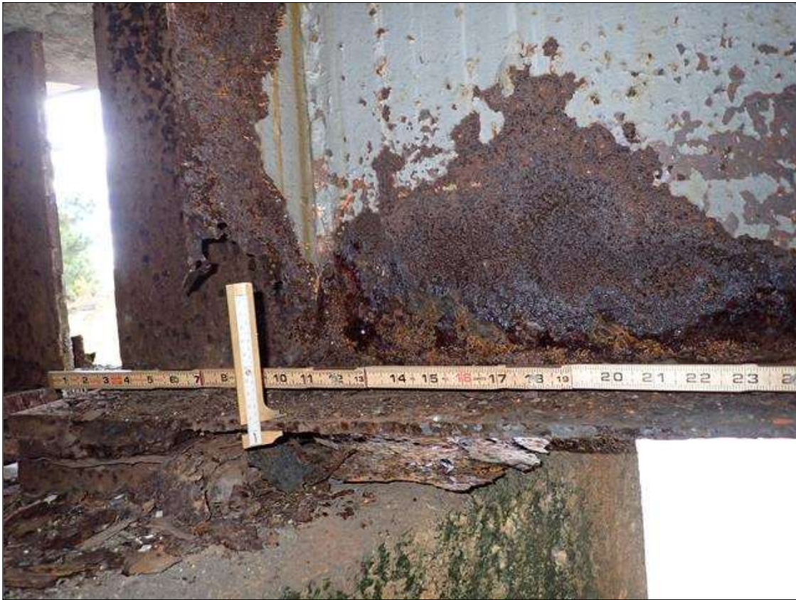
Span 4 Beam 1: PAR: CORROSION ALONG BOTH FACES OF WEB AND BOTTOM FLANGE UP TO 68 INCH LONG X UP TO 20 INCH HIGH DOWN TO 1/4 INCH RESIDUAL WEB WITH PIN HOLES BEHIND STIFFENER AND 52 INCH LONG X 10 INCH WIDE DOWN TO 5/16 INCH RESIDUAL BOTTOM FLANGE EXTENDING FROM BENT 3
