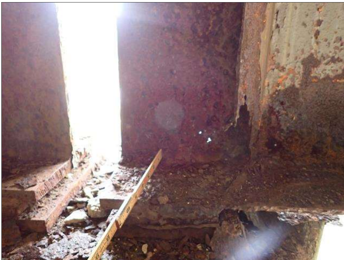
Span 4 Beam 1 - Near Bearing: PAR: MISSING ANCHOR ROD ON BOTH SIDES
