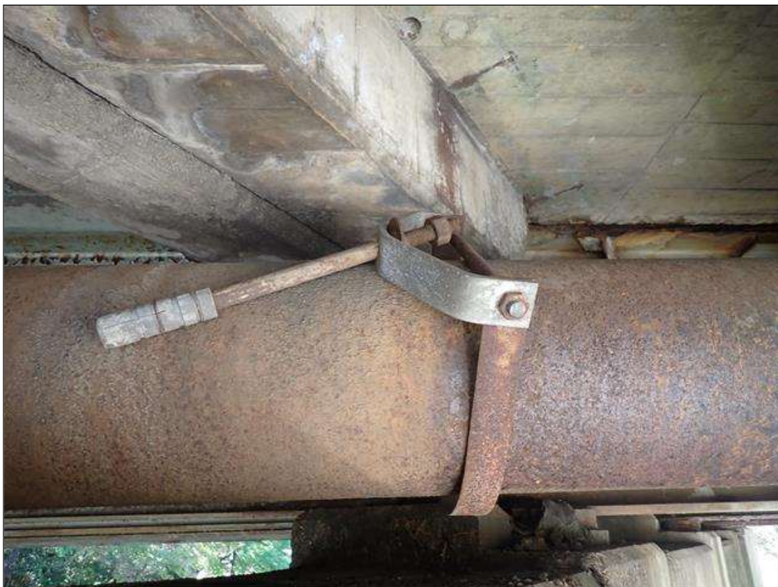
APPROXIMATELY 5 BROKEN UTILITY HANGERS IN VARIOUS LOCATIONS
