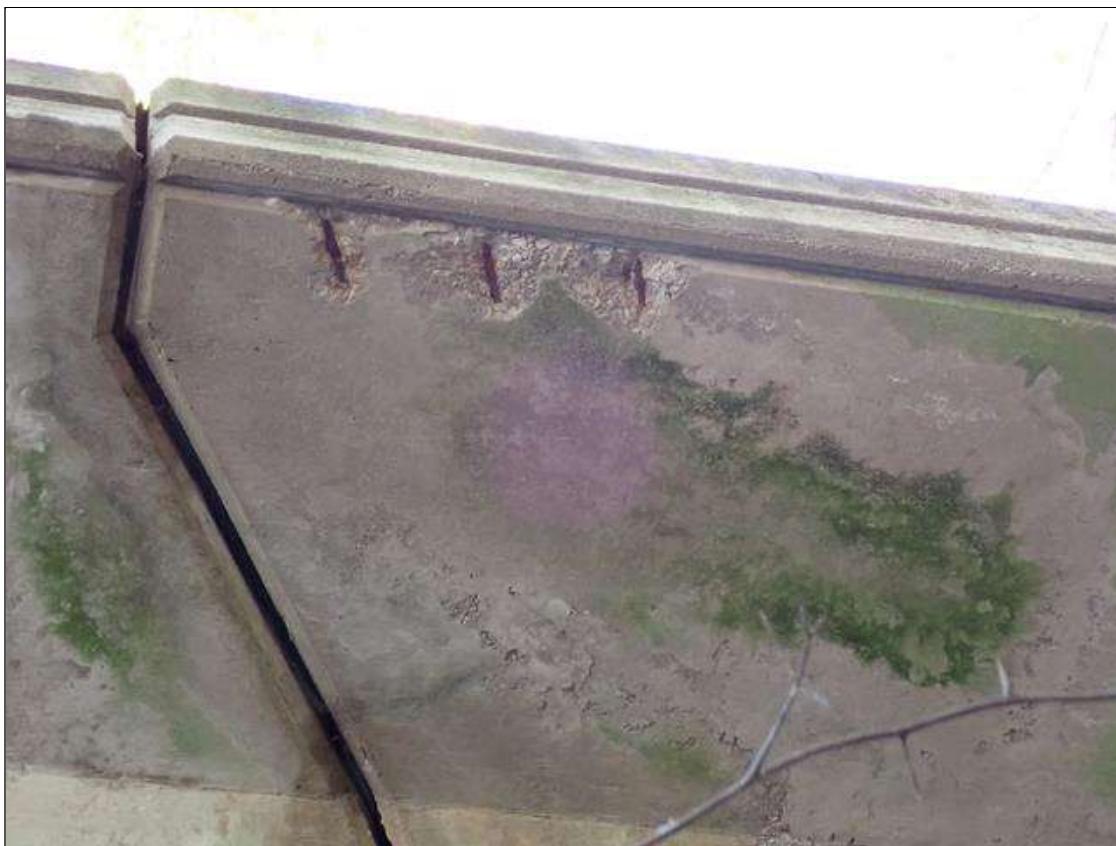
Span 1 Deck: (3) SPALLS UP TO 6 INCH X 6 INCH X 1 INCH DEEP WITH EXPOSED REBAR IN BOTTOM OF LEFT OVERHANG AT FAR END
