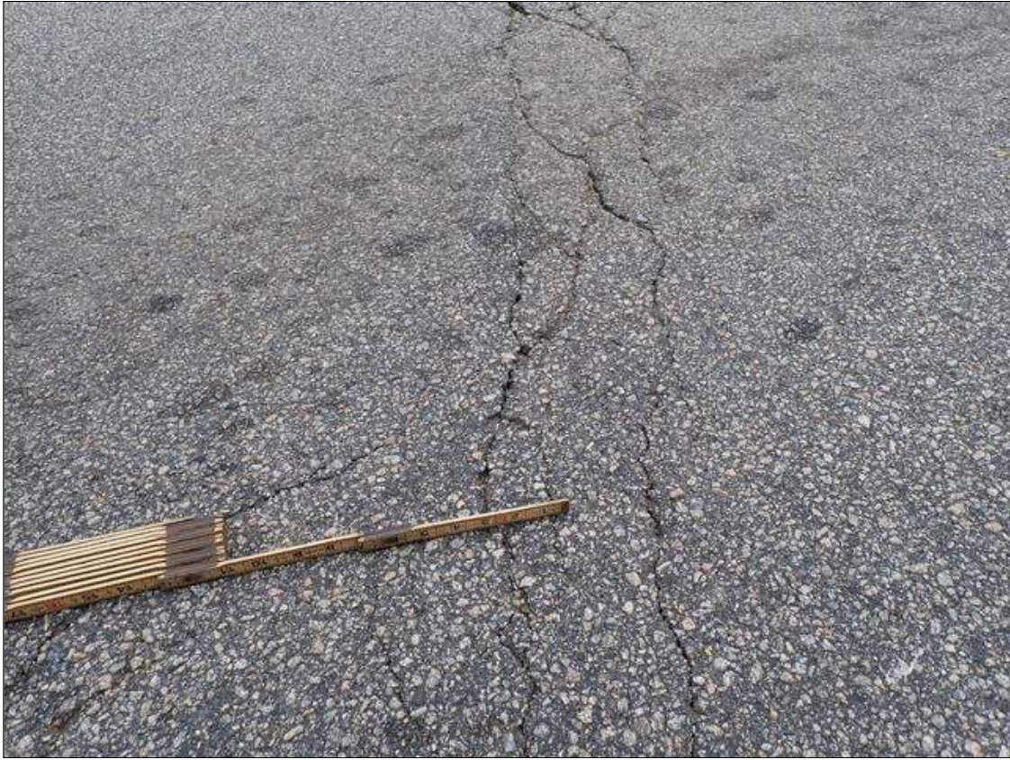
Span 1 Wearing Surface: UP TO 1/8 INCH TRANSVERSE CRACKS ALONG END BENT 1
