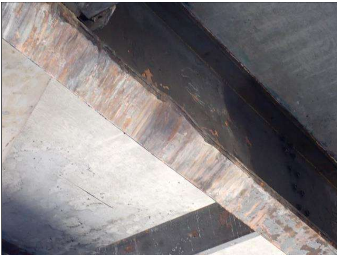
Span 3 Beam 3: UP TO 1 INCH VERTICAL DEFLECTION FROM IMPACT DAMAGE NEAR MIDSPAN
