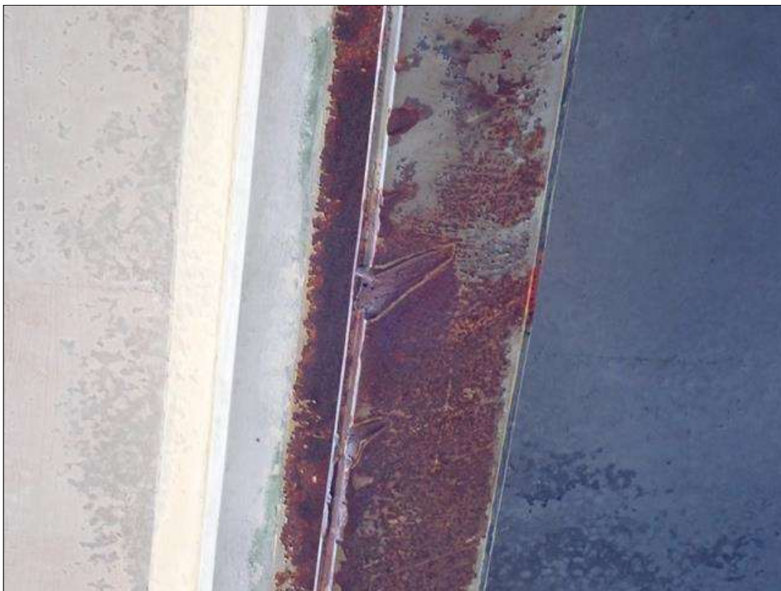
Span 2 Beam 1: PAR: IMPACT DAMAGE TO BOTTOM COVER PLATE WITH 3 INCH X 1 INCH X 1/16 INCH GOUGE AND UP TO 1/2 INCH OF VERTICAL DEFLECTION AND 1/2 INCH OF RIGHT LATTERAL DEFLECTION LOCATED APPROXIMATELY 21 FOOT FROM BENT 1
