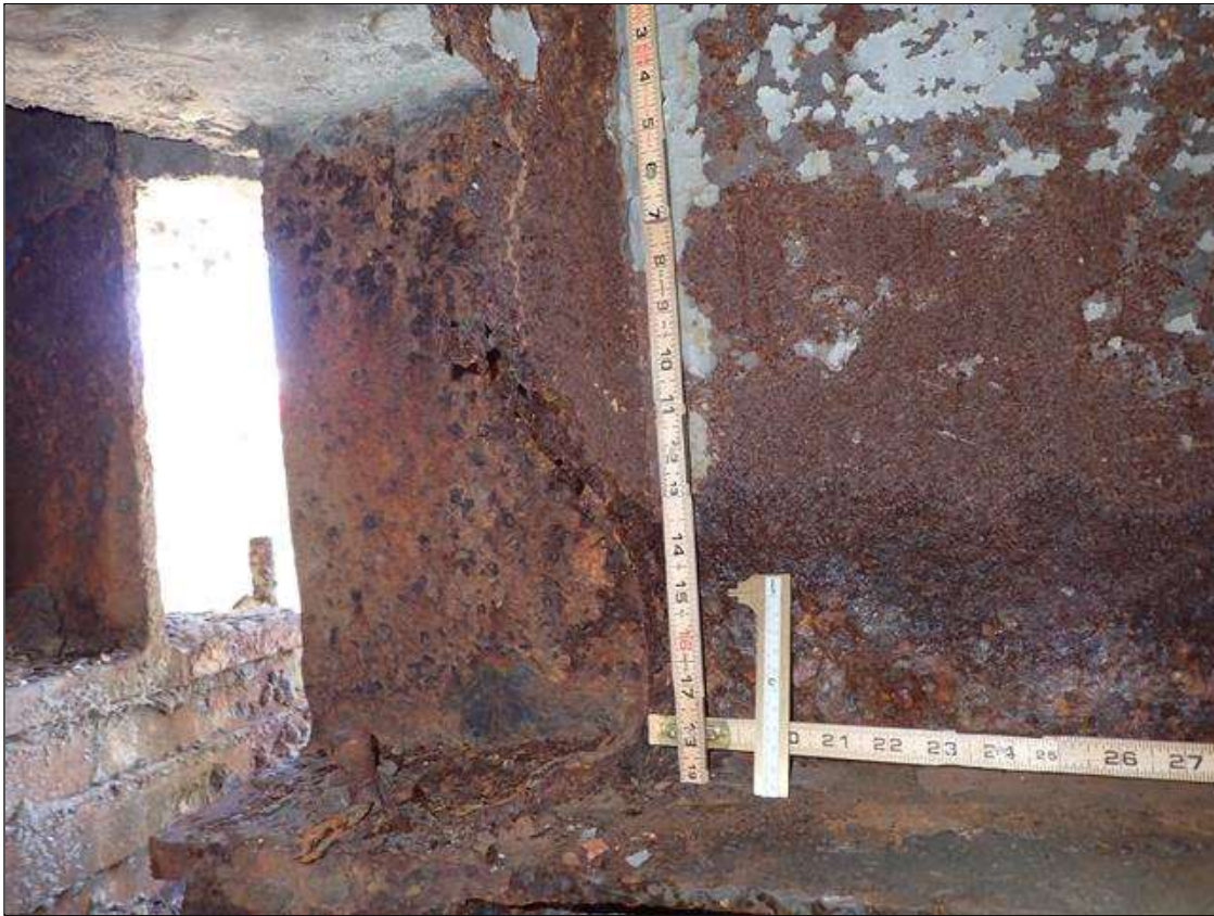
Span 2 Beam 7: PAR: CORROSION THROUGHOUT VERTICAL STIFFENER WITH 15 INCH X 5 INCH LOSS OF SECTION ON LEFT SIDE AT BENT 2 BEARING
