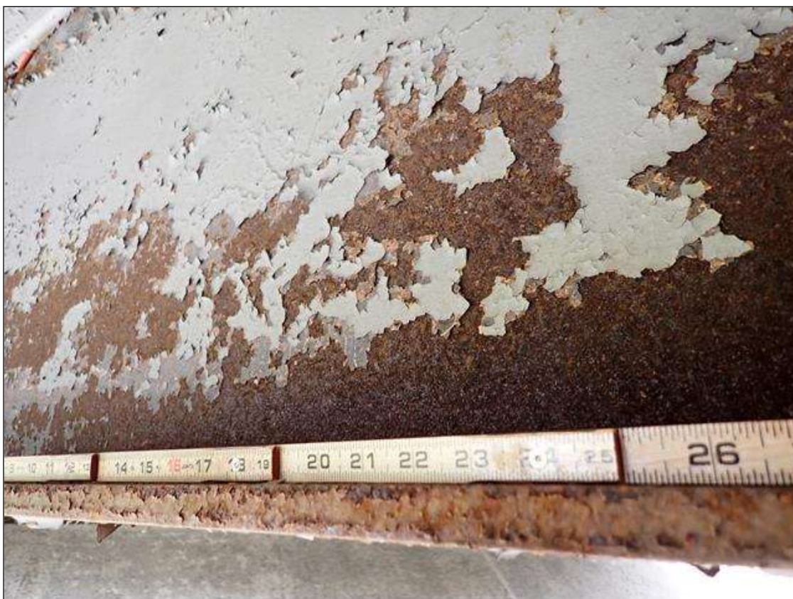
Span 4 Beam 2: AREAS OF SURFACE CORROSION THROUGHOUT
