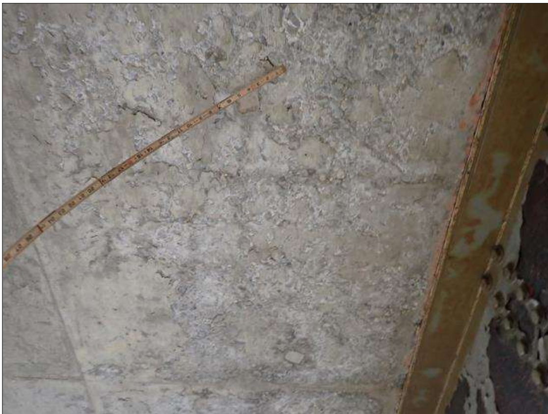
Span 1 Deck: AREAS OF POORLY CONSOLIDATED CONCRETE IN VARIOUS LOCATIONS IN BOTTOM OF DECK
