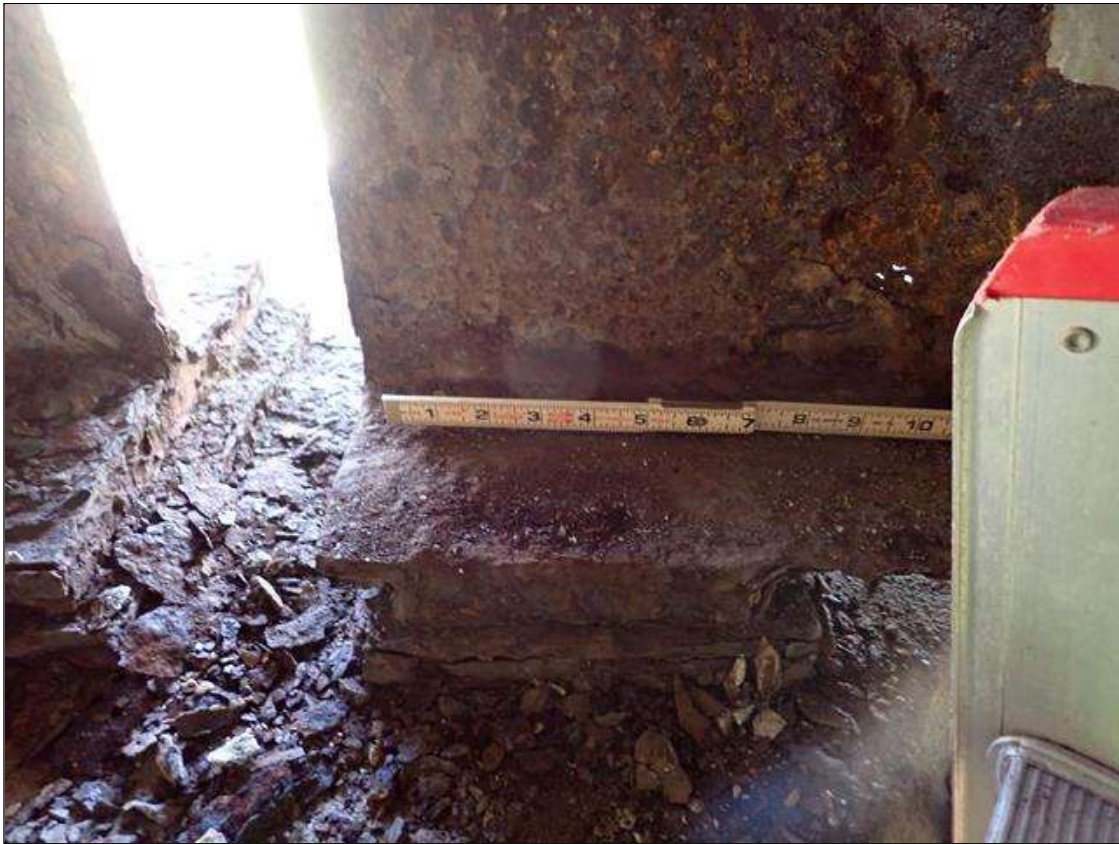
Span 1 Beam 7 - Far Bearing: PAR: MISSING ANCHOR BOLT ON LEFT SIDE
