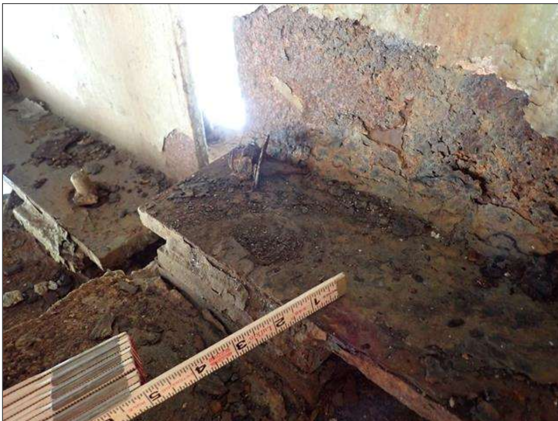
Span 4 Beam 5 - Near Bearing: PAR: MISSING ANCHOR ROD ON EAST SIDE
