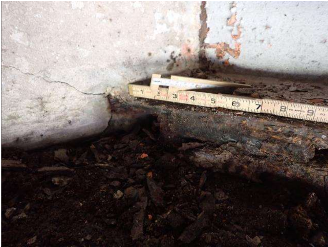
Span 1 Beam 2: PAR: CORROSION ALONG RIGHT EDGE OF BOTTOM FLANGE UP TO 10 INCH LONG X 3 INCH WIDE DOWN TO 5/8 INCH RESIDUAL FLANGE EXTENDING FROM END BENT 1
