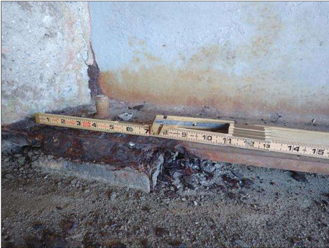
Span 1 Beam 7: PAR: CORROSION ALONG RIGHT EDGE OF BOTTOM FLANGE UP TO 10 INCH LONG X 2 INCH WIDE DOWN TO 3/16 INCH RESIDUAL FLANGE EXTENDING FROM END BENT 1
