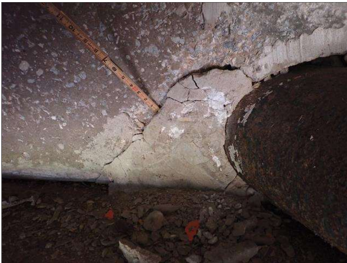
End Bent 1 Abutment: 11 INCH X 12 INCH FAILED REPAIR IN FACE OF ABUTMENT IN BAY 6 ADJACENT TO UTILITY PENETRATION
