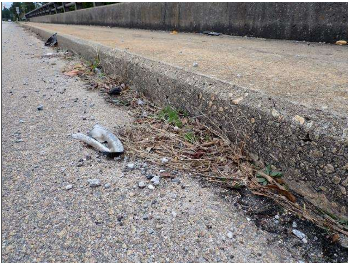
DIRT AND DEBRIS ACCUMULATION ALONG BOTH SHOULDERS
