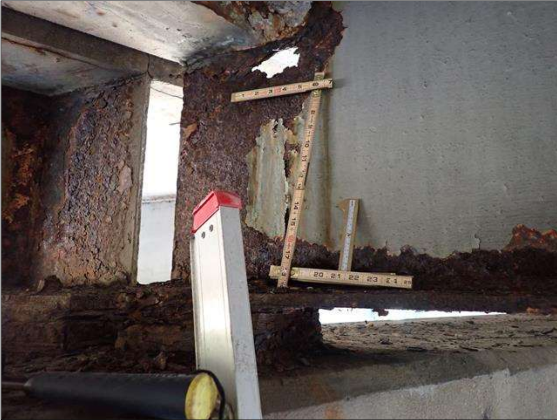
Span 1 Beam 5: PAR: CORROSION ALONG BOTH FACES OF WEB AND BOTTOM FLANGE UP TO 12 INCH LONG X 20 INCH HIGH DOWN TO KNIFES EDGE RESIDUAL WEB WITH 4 INCH X 2 INCH HOLE AT END DIAPHRAGM AND 38 INCH LONG X 10 INCH WIDE DOWN TO 5/8 INCH INCH RESIDUAL BOTTOM FLANGE EXTENDING FROM BENT 1
