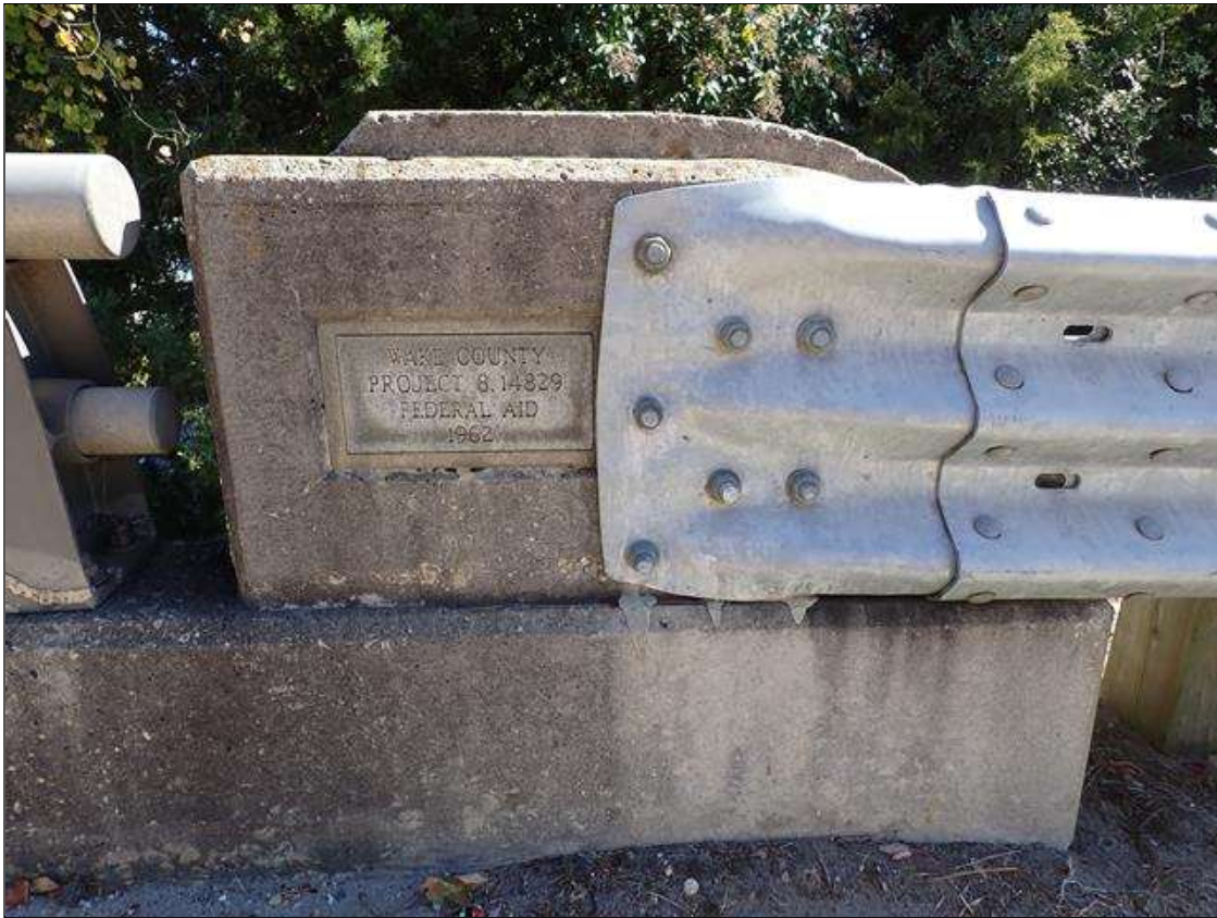
GUARDRAIL TO BARRIER RAIL CONNECTION AT SOUTHEAST CORNER, SOUTHWEST AND NORTHWEST SIMILAR
