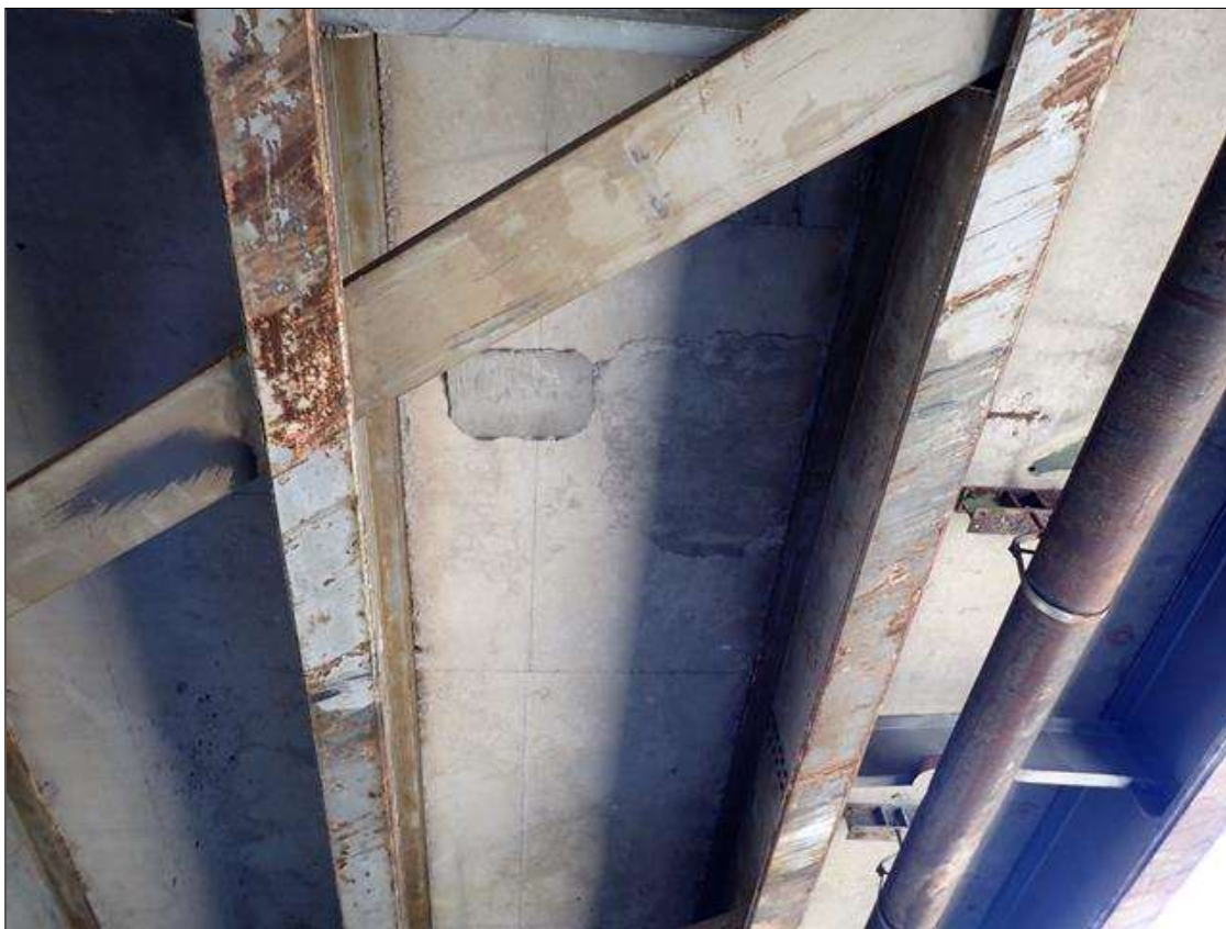
Span 3 Deck: 20 SQUARE FEET PATCHING TO UNDERSIDE OF DECK IN BAY 5, AT MIDSPAN.
