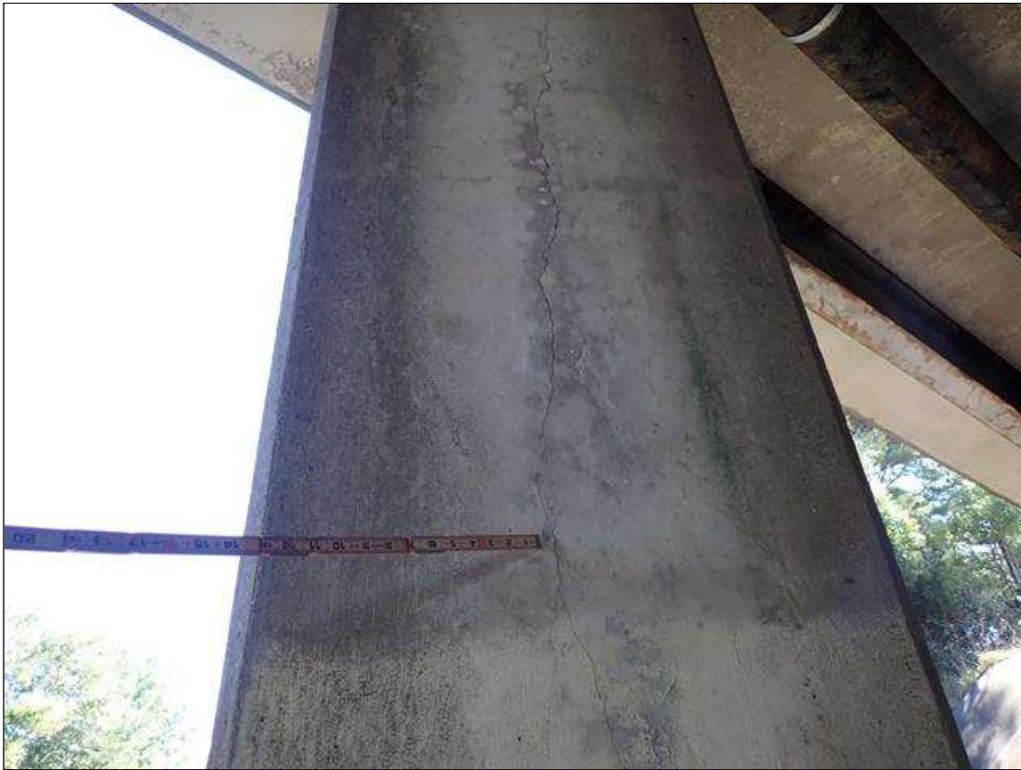
Bent 1 Pile 4: UP TO 1/16 INCH VERTICAL CRACK IN LEFT FACE OF COLUMN FOM BOTTOM OF CAP TO GROUND LINE
