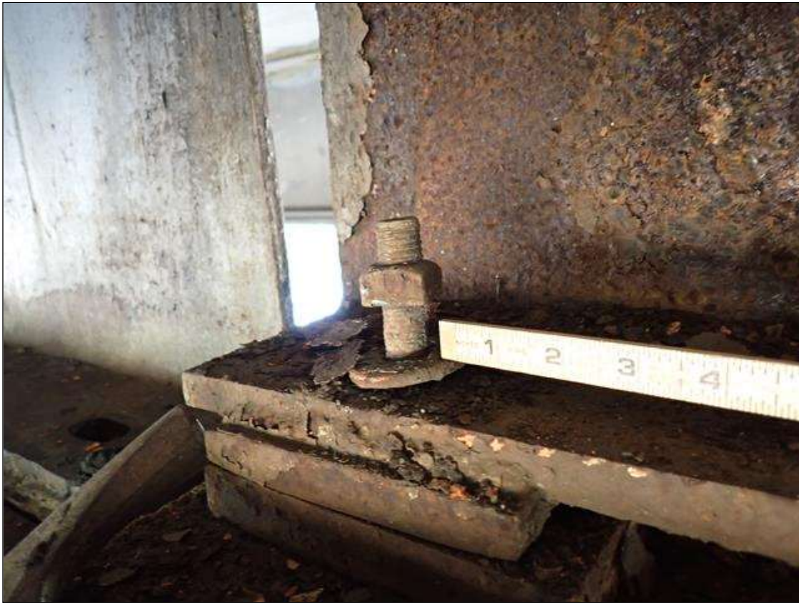
Span 4 Beam 6 - Near Bearing: ANCHOR NUT IS NOT FULLY TIGHT ON THE EAST SIDE.
