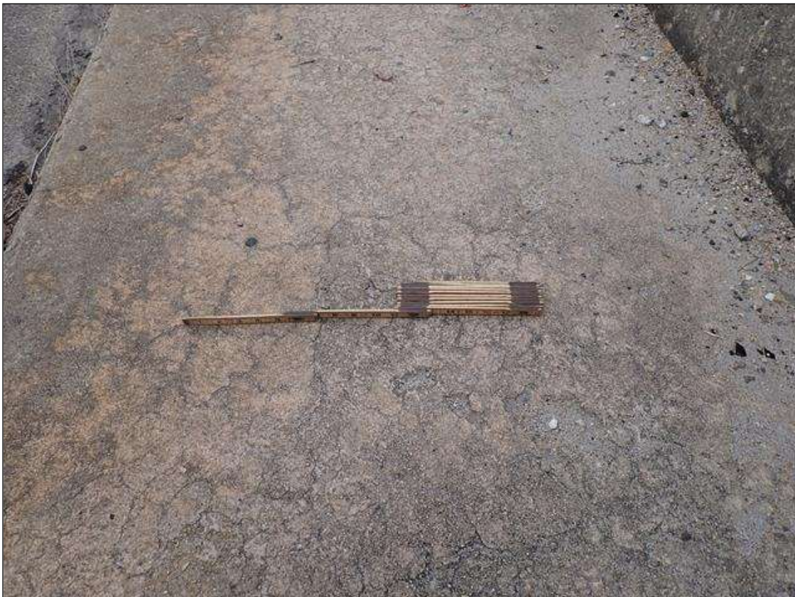
UP TO 1/16 INCH LONGITUDINAL CRACKS AND HAIRLINE MAP CRACKING IN TOP OF SIDEWALKS IN VARIOUS LOCATIONS THROUGHOUT
