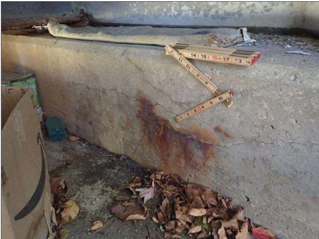
End Bent 1 Cap 1: UP TO 1/16 INCH HORIZONTAL CRACK AND HAIRLINE MAP CRACKING WITH EFFLORESCENCE AND RUST STAINING IN FACE OF CAP AT LEFT END
