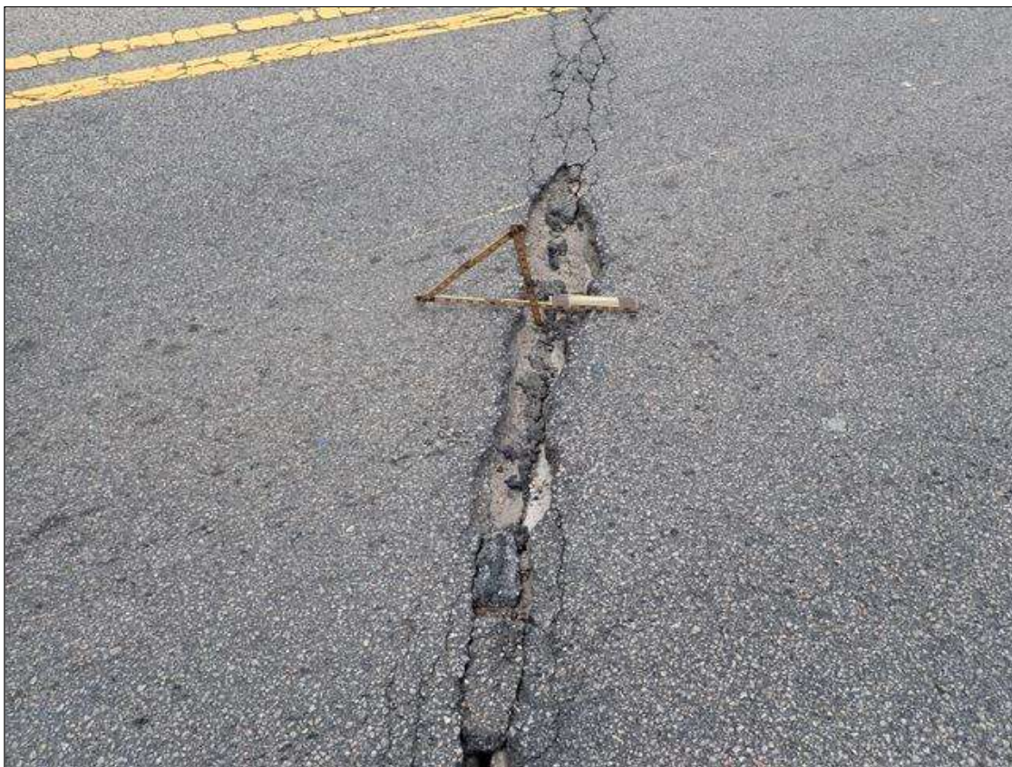
Span 3 Wearing Surface: PAR: 96 INCH LONG X 8 INCH WIDE X 3 INCH DEEP POTHOLE IN FAILED REPAIR IN CENTER OF NORTHBOUND LANE ABOVE BENT 2
