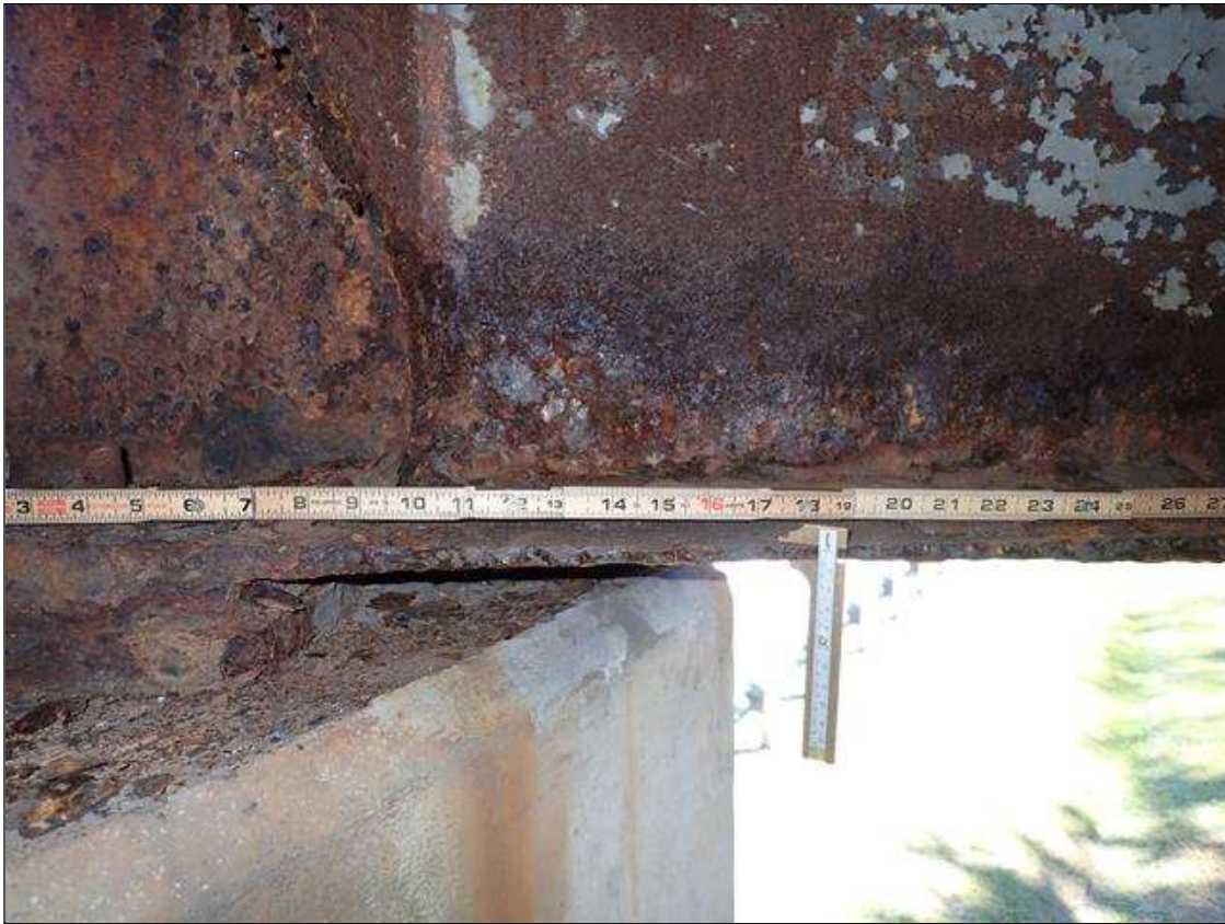
Span 2 Beam 7: PAR: CORROSION ALONG BOTH FACES OF WEB AND BOTTOM FLANGE UP TO 52 INCH LONG X 20 INCH HIGH DOWN TO 1/2 INCH RESIDUAL WEB AND 36 INCH LONG X 10 INCH WIDE DOWN TO 5/16 INCH RESIDUAL BOTTOM FLANGE EXTENDING FROM BENT 2
