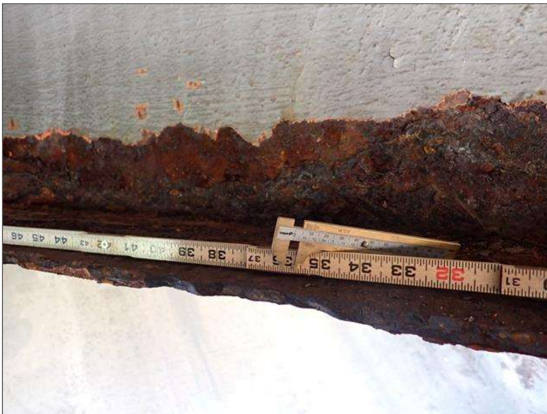
Span 1 Beam 4: PAR: CORROSION ALONG BOTH FACES OF WEB AND BOTTOM FLANGE UP TO 14 INCH LONG X 24 INCH HIGH DOWN TO 1/4 INCH RESIDUAL WEB AND 58 INCH LONG X 10 INCH WIDE DOWN TO 5/16 INCH RESIDUAL BOTTOM FLANGE EXTENDING FROM BENT 1
