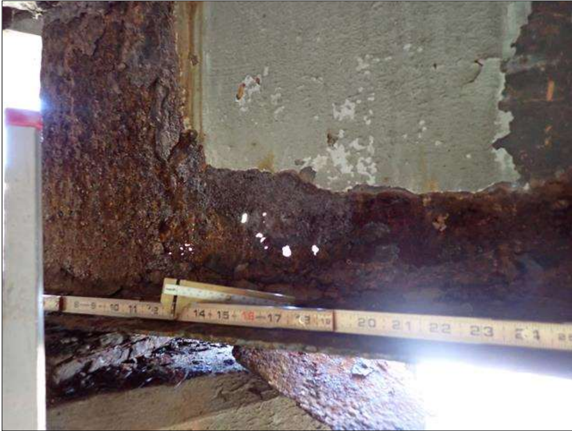
Span 1 Beam 7: PAR: CORROSION ALONG BOTH FACES OF WEB AND BOTTOM FLANGE UP TO 36 INCH LONG X UP TO 21 INCH HIGH DOWN TO KNIFE EDGE RESIDUAL WEB WITH 8 INCH X 3 INCH AREA OF UP TO 1/2 INCH DIAMETER HOLES IN WEB AND 36 INCH LONG X 10 INCH WIDE DOWN TO 1/8 INCH RESIDUAL BOTTOM FLANGE EXTENDING FROM BENT 1
