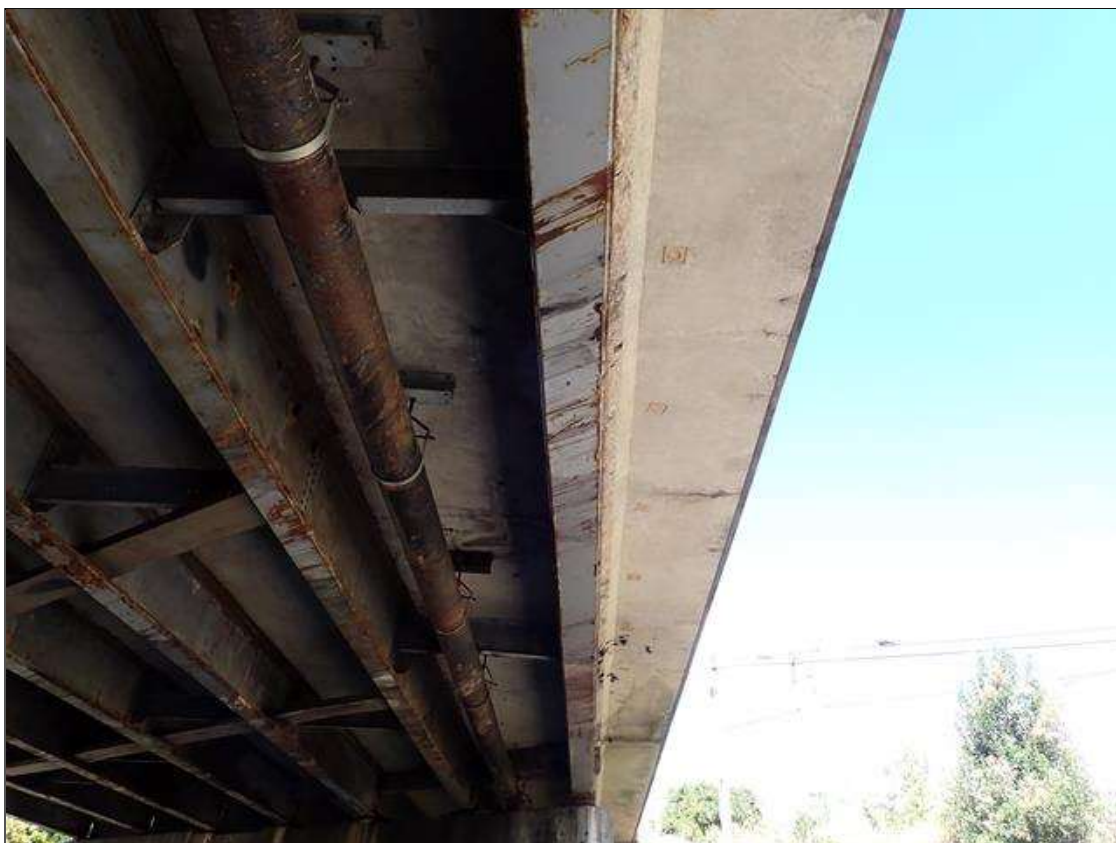
Span 3 Beam 7: 30 FOOT OF IMPACT DAMAGE WITH UP TO 1/16 INCH GOUGING THROUGHOUT (BEAM STRUCK BY TRACKER TRAILER DURING INSPECTION, DAMAGE INSPECTION REQUESTED)
