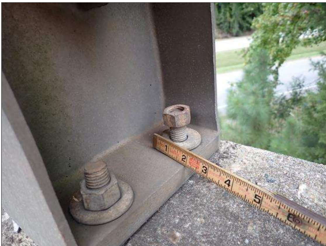
Span 1 Right Bridge Rail: LOOSE ANCHOR NUT AT SOUTHEAST CORNER OF RAIL POST 2
