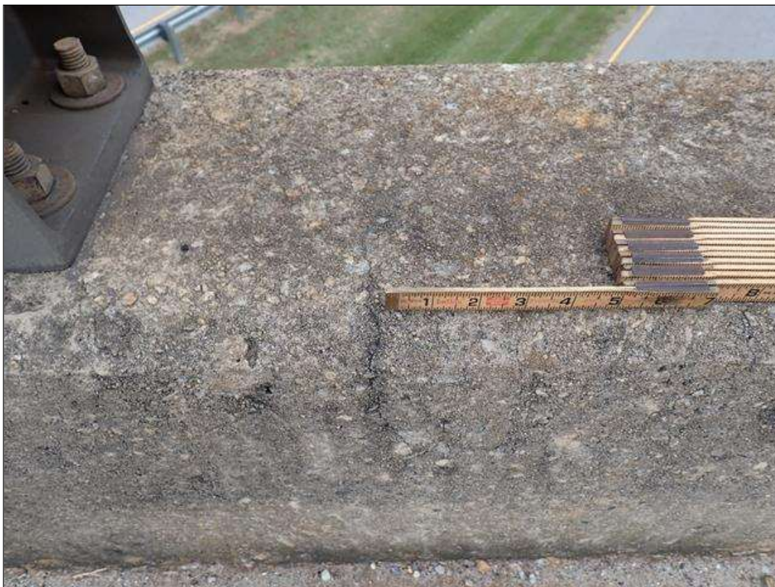
Span 2 Right Bridge Rail: UP TO 0.016 INCH TRANSVERSE AND VERTICAL CRACKS IN TOP AND BOTH FACES OF PARAPET IN VARIOUS LOCATIONS
