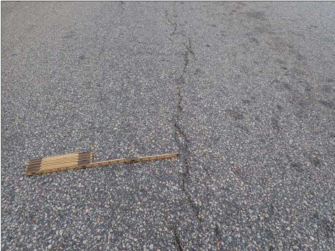
Span 1 Wearing Surface: INTERMITTENT LONGITUDINAL AND TRANSVERSE CRACKING (UP TO 1/4 INCH) THROUGHOUT ASPHALT WEARING SURFACE.
