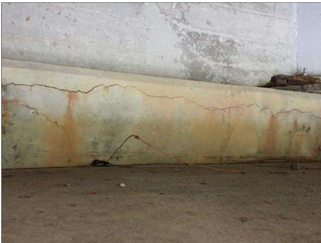
End Bent 2 Cap 1: UP TO 1/8 INCH HORIZONTAL CRACKS WITH RUST STAINING IN FACE OF CAP FROM BEAM 2 TO BEAM 3
