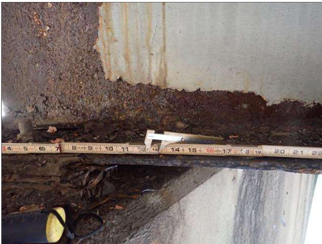
Span 1 Beam 6: PAR: CORROSION ALONG BOTH FACES OF WEB AND BOTTOM FLANGE UP TO 13 INCH LONG X 19 INCH HIGH DOWN TO 1/2 INCH RESIDUAL WEB AND 40 INCH LONG X 10 INCH WIDE DOWN TO 5/8 INCH RESIDUAL BOTTOM FLANGE EXTENDING FROM BENT 1
