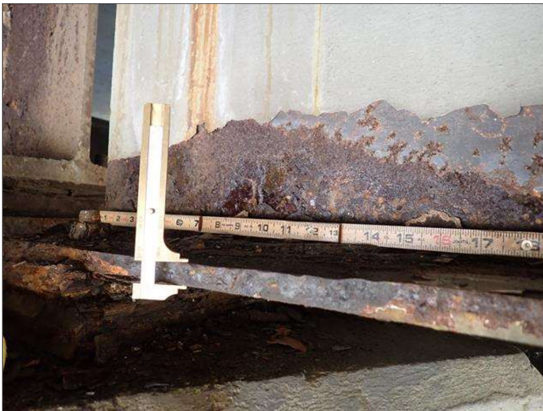
Span 3 Beam 5: PAR: CORROSION ALONG BOTH FACES OF WEB AND BOTTOM FLANGE UP TO 30 INCH LONG X 6 INCH HIGH WITH NO MEASURABLE LOSS OF SECTION IN WEB AND 17 INCH LONG X 5 INCH WIDE DOWN TO 5/8 INCH RESIDUAL BOTTOM FLANGE EXTENDING FROM BENT 2
