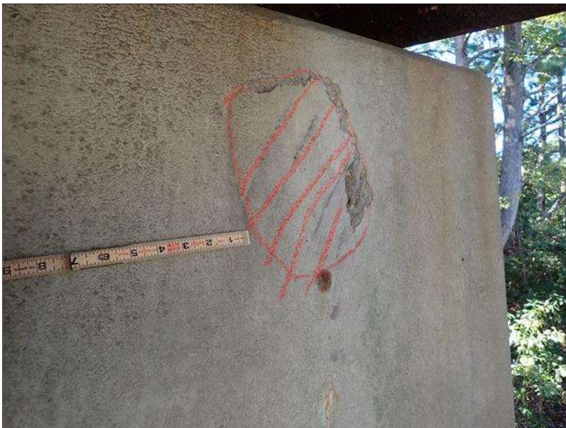
Bent 1 Cap 1: 10 INCH X 8 INCH AREA OF DELAMINATION IN SPAN 2 FACE OF CAP BENEATH BEAM 1
