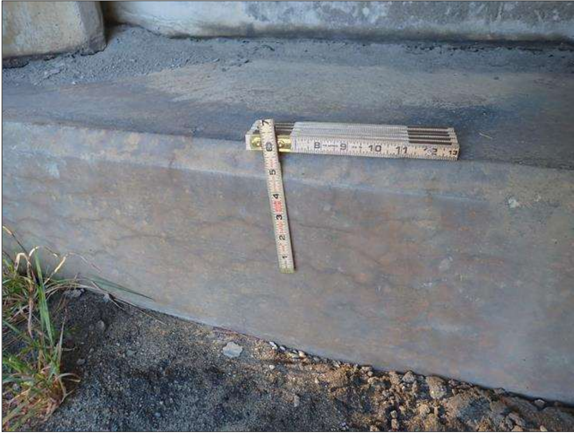
End Bent 1 Cap 1: HAIRLINE MAP CRACKING IN FACE OF CAP AT RIGHT END
