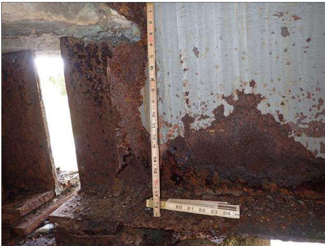
Span 4 Beam 1: PAR: CORROSION THROUGHOUT RIGHT SIDE STIFFENER DOWN TO KNIFES EDGE WITH (2) HOLES UP TO 5 INCH X 4 INCH AT BENT 3
