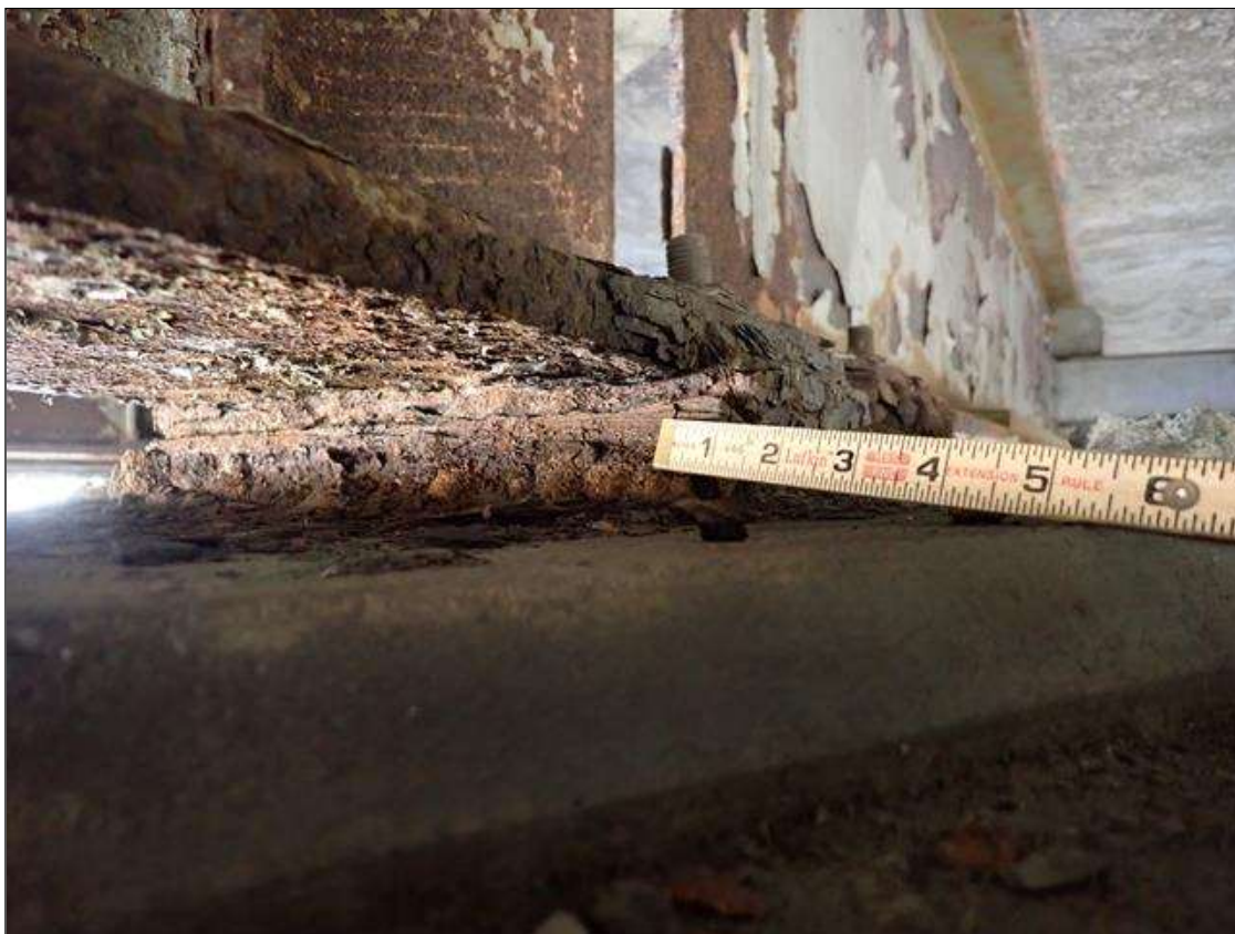
Span 2 Beam 4 - Near Bearing: CORROSION THROUGHOUT
