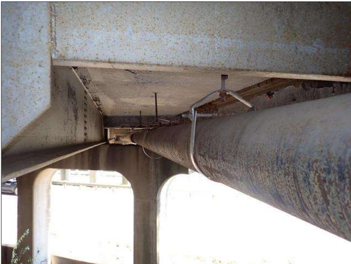
12 INCH DIAMETER DUCTILE IRON UTILITY ATTACHED TO BOTTOM OF DECK IN BAY 6
