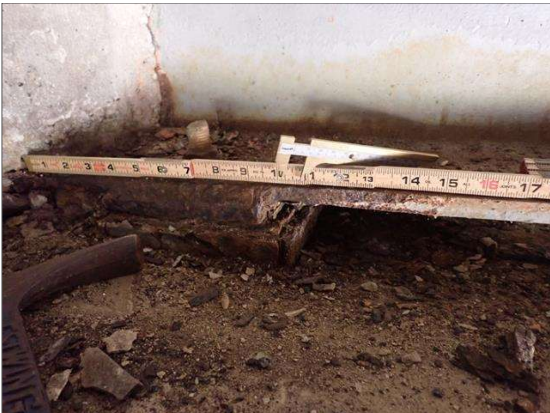
Span 1 Beam 3: PAR: CORROSION ALONG RIGHT EDGE OF BOTTOM FLANGE UP TO 12 INCH LONG X 4 INCH WIDE DOWN TO 1/2 INCH INCH RESIDUAL FLANGE EXTENDING FROM END BENT 1
