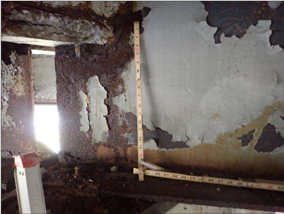
Span 1 Beam 3: PAR: CORROSION ALONG BOTH FACES OF WEB AND BOTTOM FLANGE UP TO 12 INCH LONG X 20 INCH HIGH DOWN TO 5/16 INCH RESIDUAL WEB AND 35 INCH LONG X 10 INCH WIDE DOWN TO 1/2 INCH RESIDUAL BOTTOM FLANGE AT BENT 1
