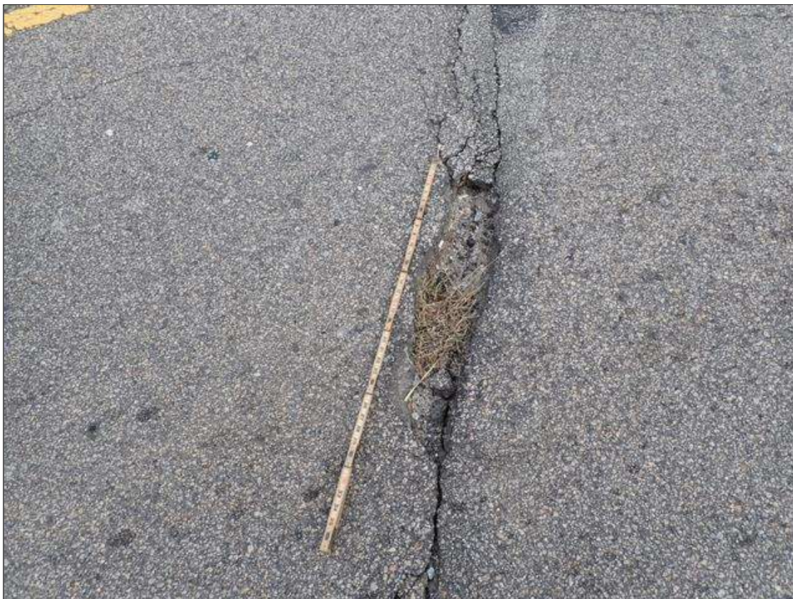
Span 4 Wearing Surface: PAR: 28 INCH X 8 INCH X 3 INCH DEEP POTHOLE IN CENTER OF SOUTHBOUND LANE ABOVE BENT 3
