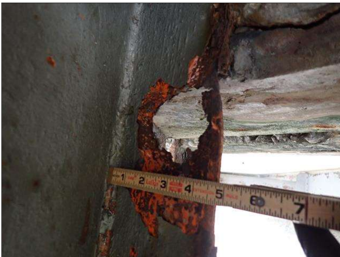
Span 3 Beam 1: PAR: CORROSION THROUGHOUT RIGHT SIDE STIFFENER DOWN TO KNIFES EDGE WITH (2) HOLES UP TO 4 INCH X 4 INCH AT BENT 3
