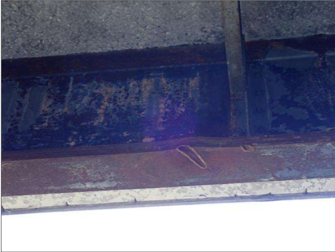
Span 2 Beam 7: PAR: IMPACT DAMAGE TO BOTTOM COVER PLATE WITH 1 1/2 INCH X 1/2 INCH X 1/16 INCH GOUGE AND 11 INCH LONG BROKEN WIELD WITH UP TO 1 INCH OF VERTICAL DEFLECTION LOCATED APPROXIMATELY 21 FOOT FROM BENT 1
