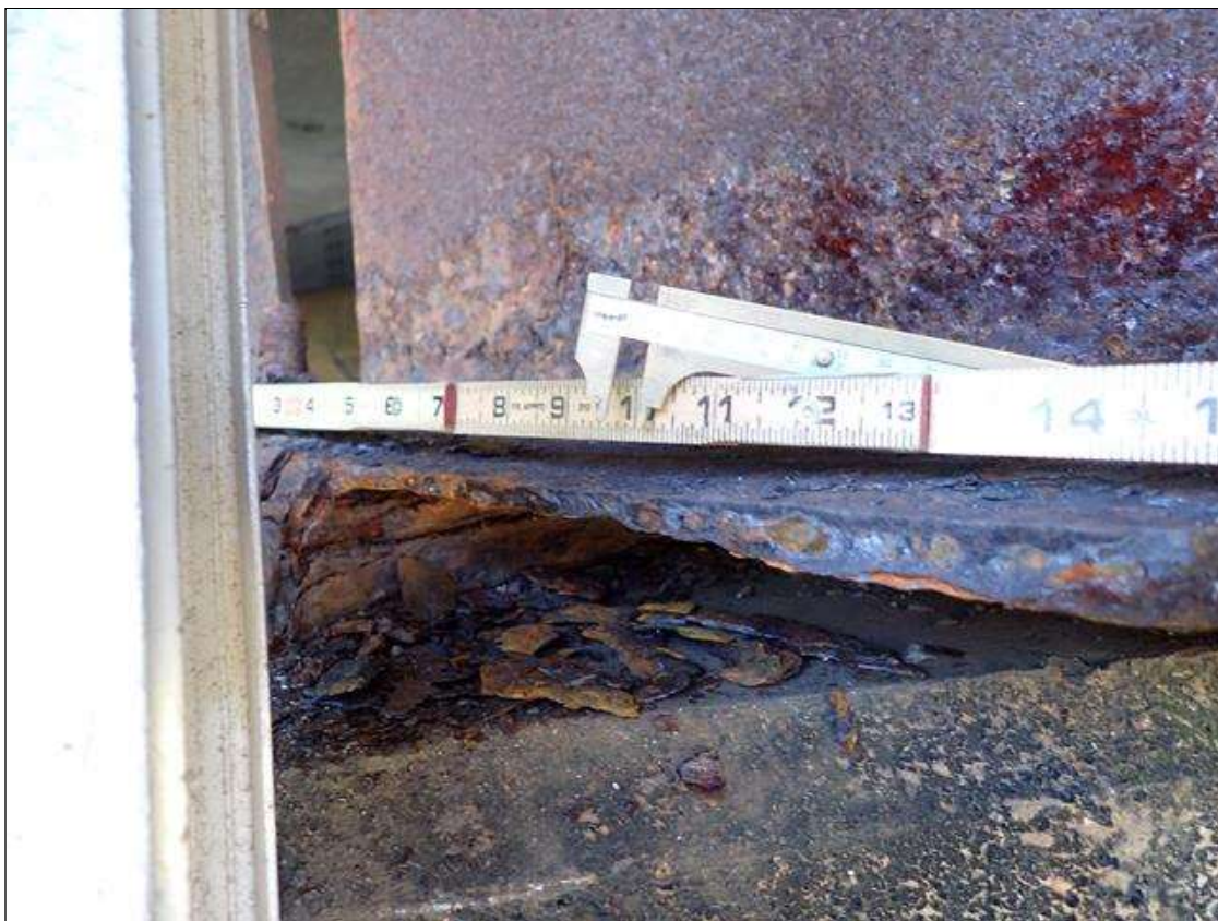
Span 2 Beam 7: PAR: CORROSION ALONG BOTH FACES OF WEB AND BOTTOM FLANGE UP TO 18 INCH LONG X 20 INCH HIGH WITH NO MEASURABLE LOSS OF SECTION IN WEB AND 23 INCH LONG X 10 INCH WIDE DOWN TO 5/16 INCH RESIDUAL BOTTOM FLANGE EXTENDING FROM BENT 1
