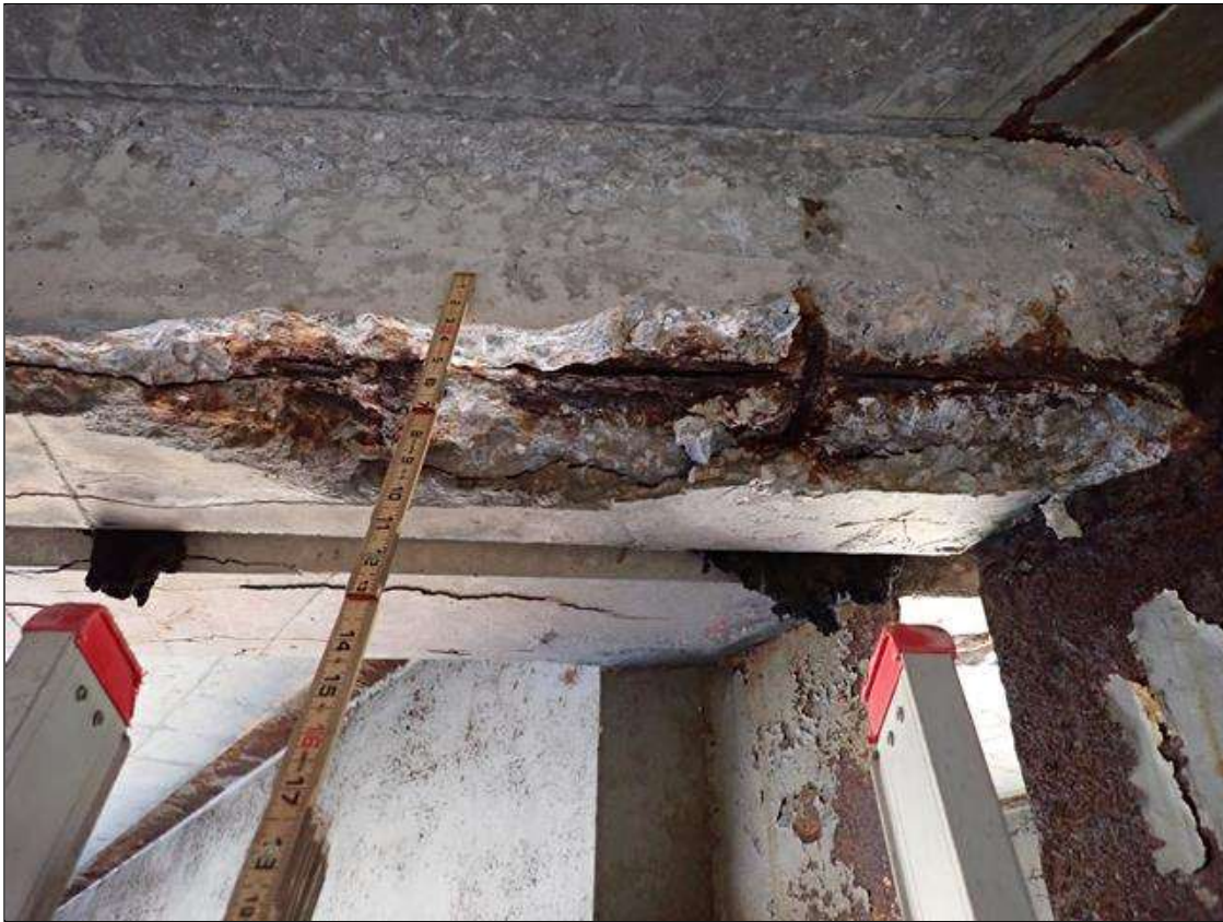
Span 1 Beam 2: 38 INCH LONG X 7 INCH WIDE X 1 INCH DEEP SPALL WITH EXPOSED REBAR IN END DIAPHRAGM ADJACENT TO BEAM 3
