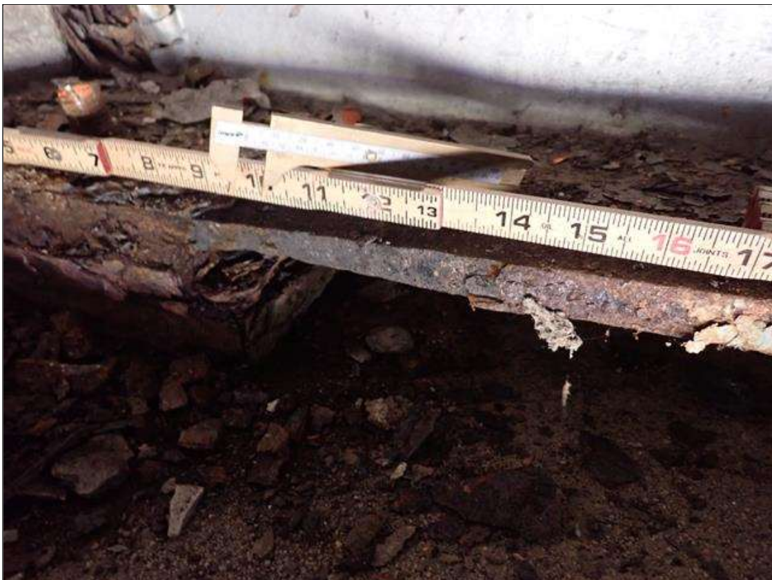
Span 1 Beam 1: PAR: CORROSION ALONG RIGHT EDGE OF BOTTOM FLANGE UP TO 16 INCH LONG X 4 INCH WIDE DOWN TO 5/8 INCH RESIDUAL FLANGE EXTENDING FROM END BENT 1
