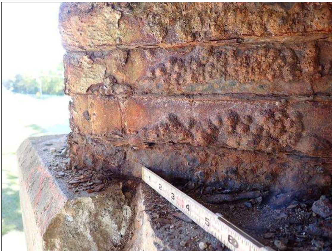
Span 3 Beam 7 - Near Bearing: AREA OF DELAMINATION IN SPAN 3 FACE OF CAP BENEATH BEAM 7 NEAR BEARING WITH APPROXIMATELY 3 INCH X 3 INCH LOSS OF BEARING
