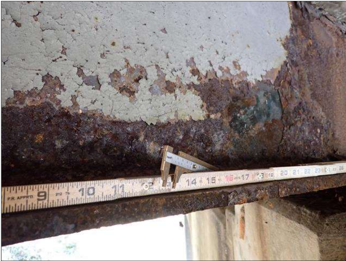
Span 4 Beam 4: PAR: CORROSION ALONG BOTH FACES OF WEB AND BOTTOM FLANGE UP TO 47 INCH LONG X 18 INCH HIGH DOWN TO 1/2 INCH RESIDUAL WEB AND 52 INCH LONG X 10 INCH WIDE DOWN TO 5/8 INCH RESIDUAL BOTTOM FLANGE EXTENDING FROM BENT 3
