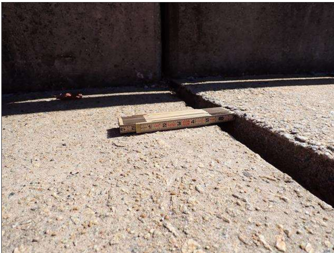
SAG ALONG RIGHT SIDE OF SPAN 3 DECK AND RAIL ABOVE BEAM 7 WITH VERTICAL DEFLECTION OF DECK AND SIEWALK AT BENTS 2 AND 3
