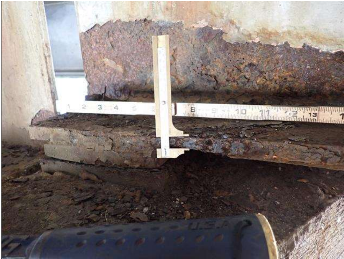
Span 4 Beam 5: PAR: CORROSION ALONG BOTH FACES OF WEB AND BOTTOM FLANGE UP TO 16 INCH LONG X 6 INCH HIGH WITH NO MEASURABLE LOSS OF SECTION IN WEB AND 14 INCH LONG X 4 INCH WIDE DOWN TO 1/2 INCH RESIDUAL BOTTOM FLANGE EXTENDING FROM BENT 3
