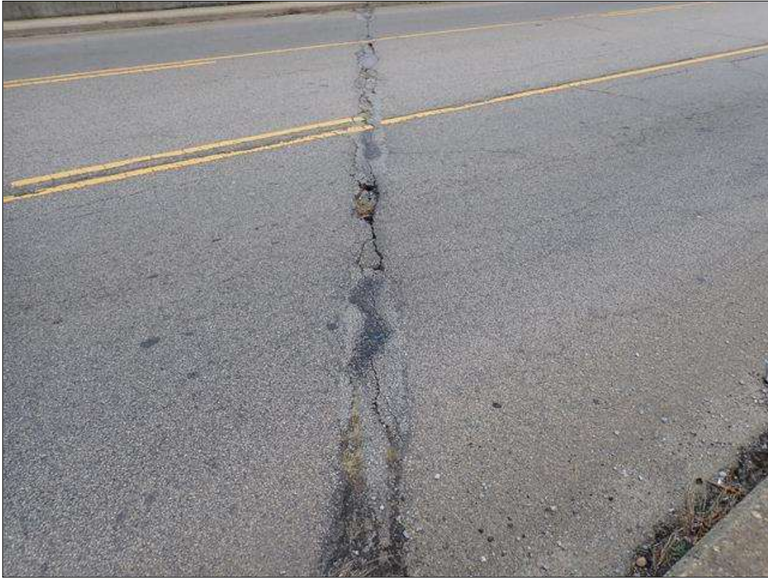
Span 4 Wearing Surface: 18 FOOT OF FAILED REPAIR PRIMARILY IN CENTER LANE ALONG BENT 3
