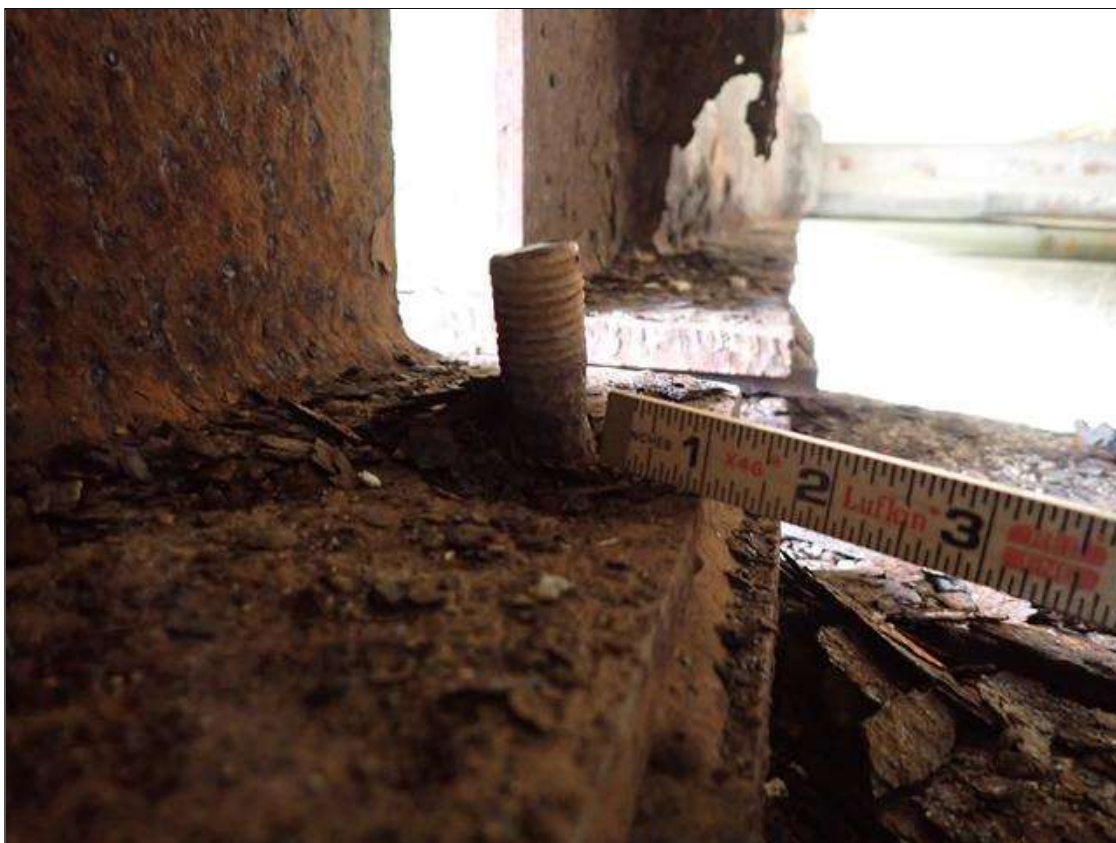
Span 3 Beam 1 - Far Bearing: PAR: MISSING ANCHOR NUT ON EAST SIDE
