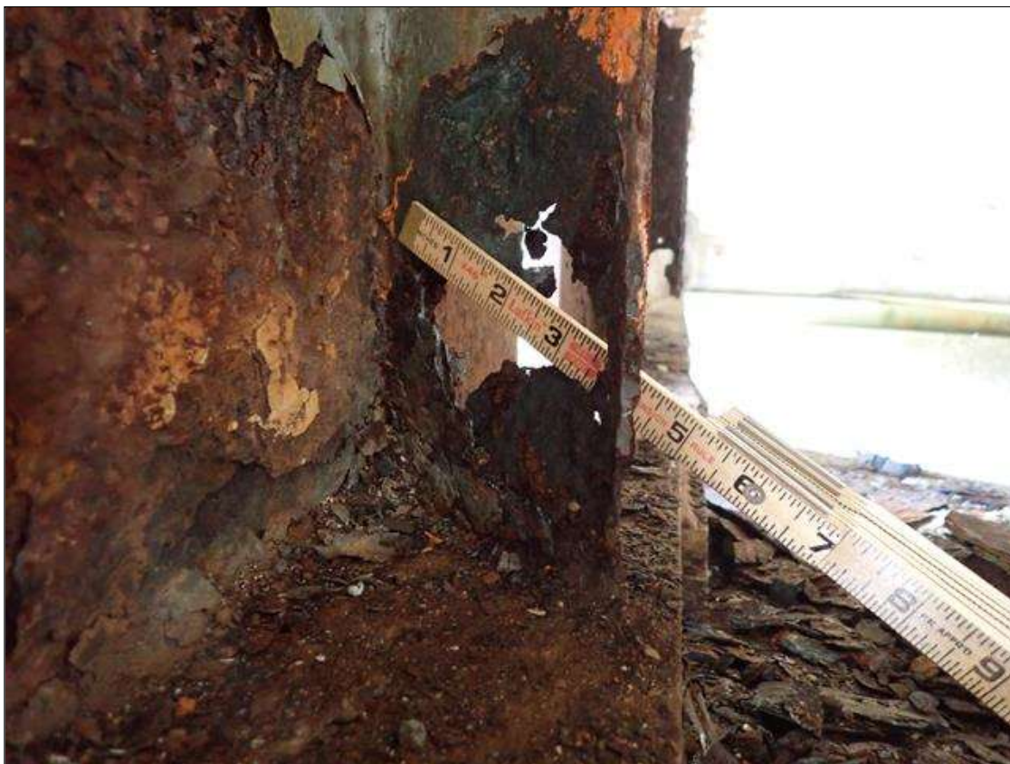
Span 3 Beam 1: PAR: CORROSION THROUGHOUT RIGHT SIDE STIFFENER DOWN TO KNIFES EDGE WITH (2) HOLES UP TO 4 INCH X 4 INCH AT BENT 3
