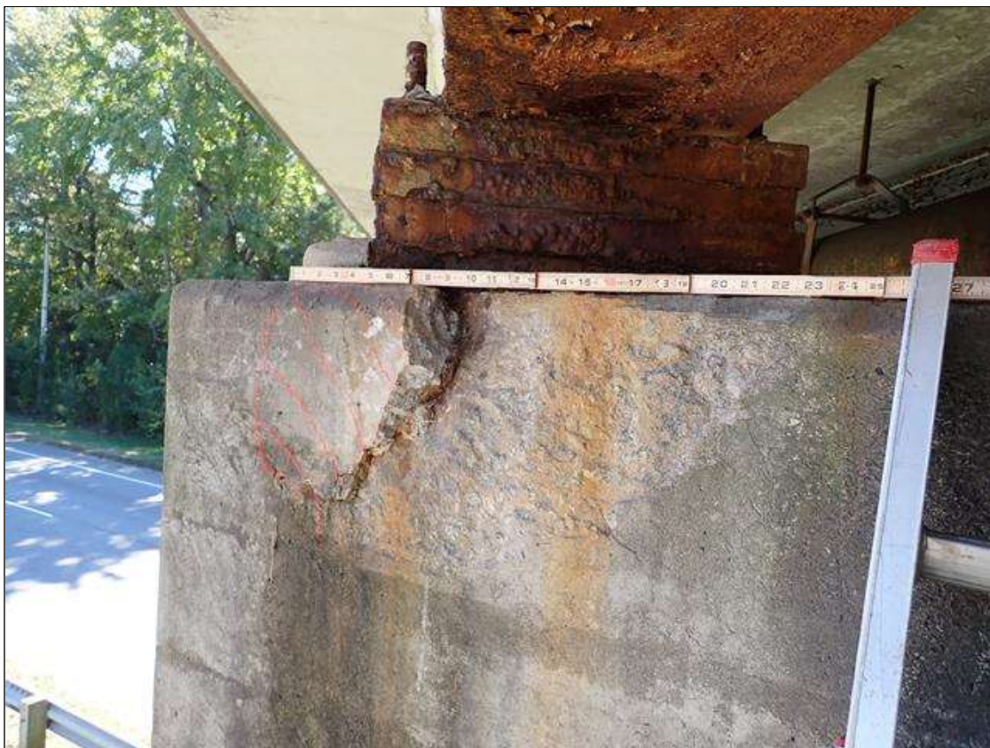
Bent 2 Cap 1: PAR: 9 INCH WIDE X 10 INCH HIGH AREA OF DELAMINATION WITH 15 INCH WIDE X 10 INCH HIGH X 3 INCH DEEP SPALL WITH EXPOSED REBAR IN TOP AND SPAN 3 FACE OF CAP BENEATH BEAM 7 BEARING
