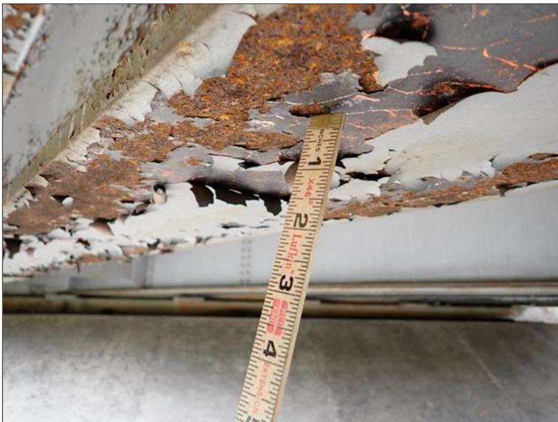
Span 4 Beam 2 - Protective System: PEELING PAINT ALONG WEB AND BOTH FLANGES IN VARIOUS LOCATIONS
