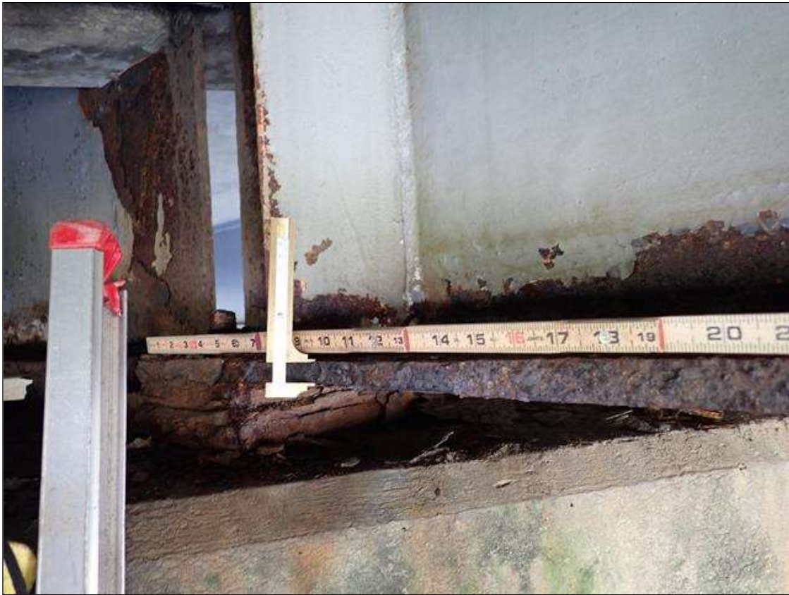
Span 2 Beam 6: PAR: CORROSION ALONG BOTH FACES OF WEB AND BOTTOM FLANGE UP TO 10 INCH LONG X 16 INCH HIGH WITH NO MEASURABLE LOSS OF SECTION IN WEB AND 17 INCH LONG X 4 INCH WIDE DOWN TO 5/8 INCH RESIDUAL BOTTOM FLANGE AT BENT 1
