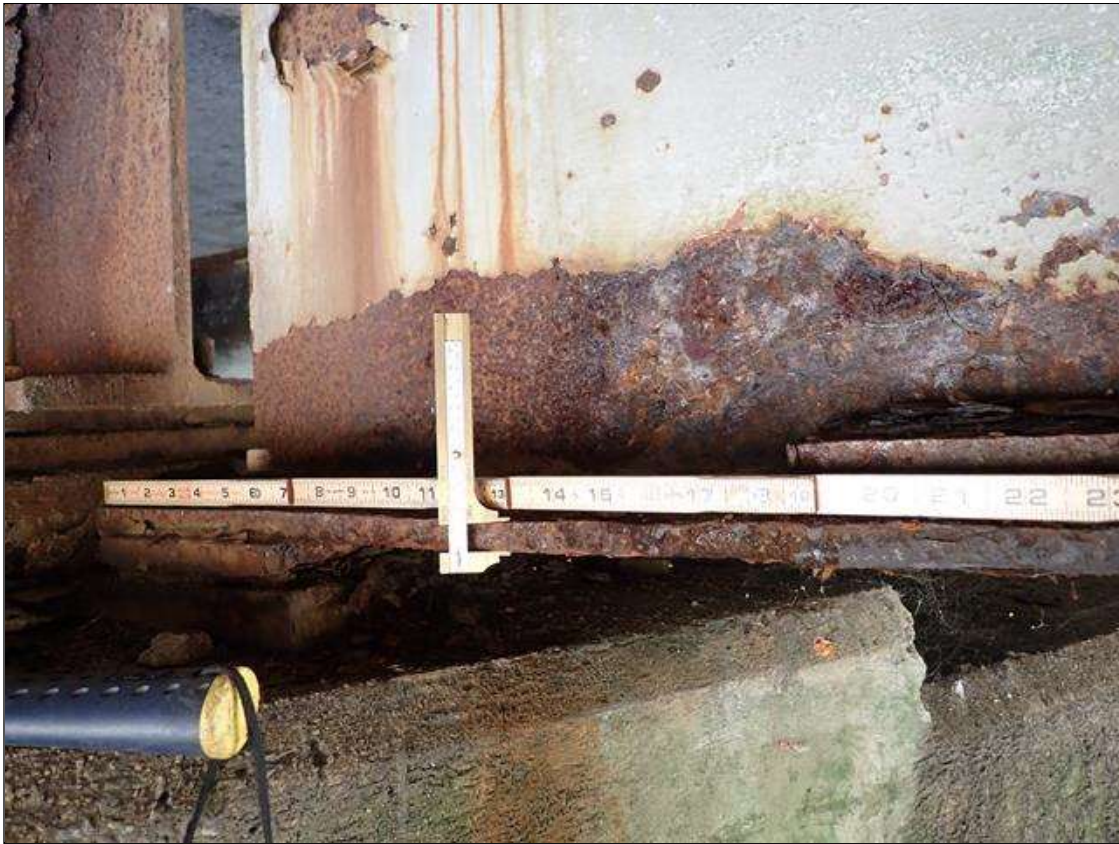
Span 3 Beam 4: PAR: CORROSION ALONG BOTH FACES OF WEB AND BOTTOM FLANGE UP TO 26 INCH LONG X 6 INCH HIGH DOWN TO 1/2 INCH RESIDUAL WEB AND 34 INCH LONG X 10 INCH WIDE DOWN TO 9/16 INCH RESIDUAL BOTTOM FLANGE EXTENDING FROM BENT 2
