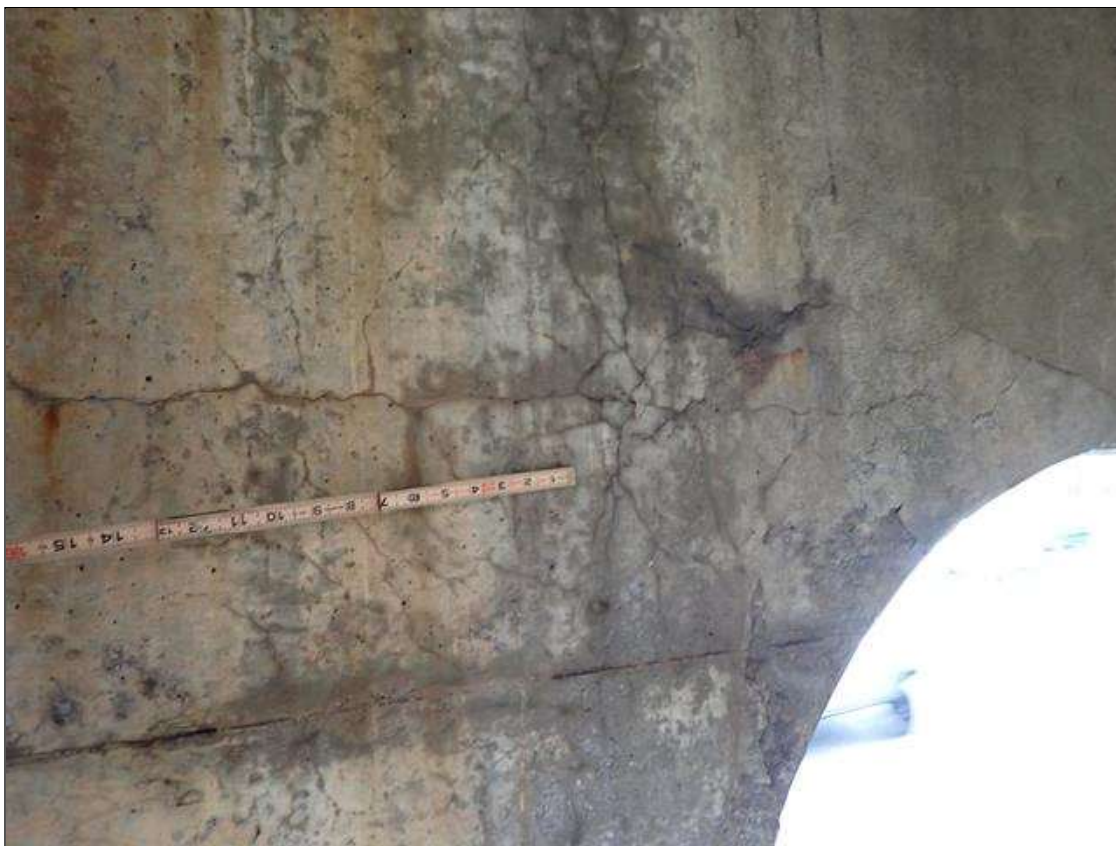
Bent 3 Cap 1: 34 INCH X 30 INCH AREA OF DELAMINATION WITH MAP CRACKING UP TO 1/16 INCH IN SPAN 4 FACE OF CAP BENEATH BEAM 5
