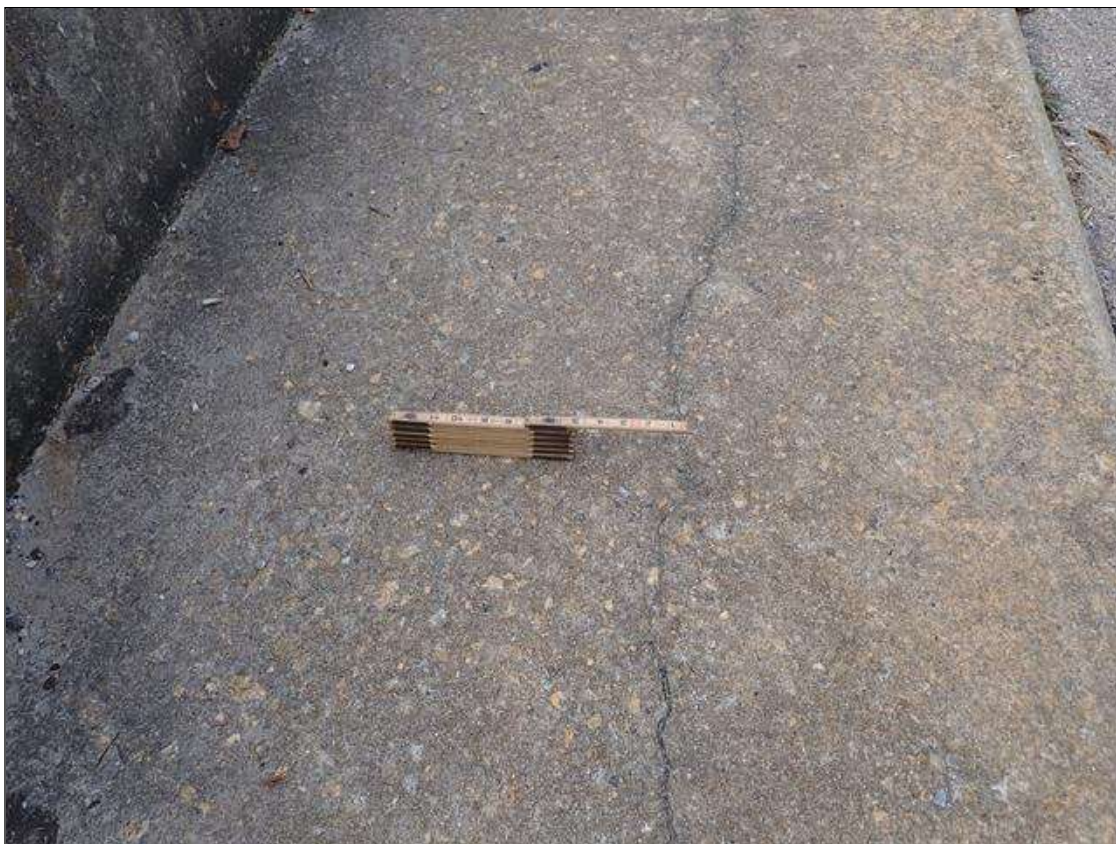
UP TO 1/16 INCH LONGITUDINAL CRACKS AND HAIRLINE MAP CRACKING IN TOP OF SIDEWALKS IN VARIOUS LOCATIONS THROUGHOUT
