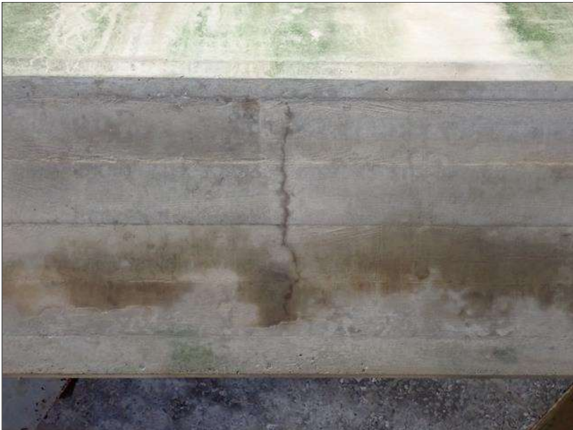
Bent 1 Cap 1: UP TO 0.05 INCH X 20 INCH TRANSVERSE CRACK IN BOTTOM OF CAP BETWEEN COLUMNS 2 AND 3
