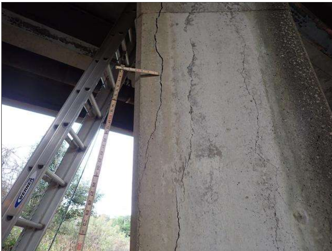
Bent 3 Pile 4: UP TO 1/8 INCH X 74 INCH LONG VERTICAL CRACKS IN LEFT FACE OF COLUMN AT BOTTOM OF CAP
