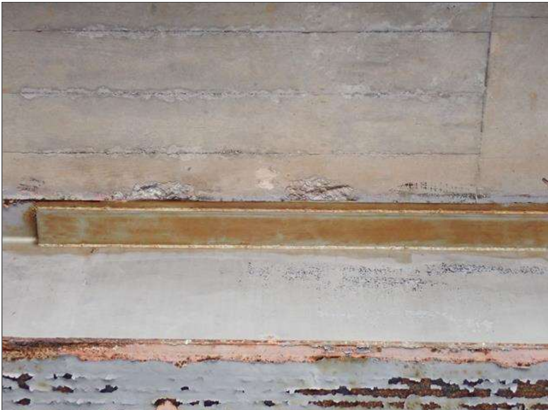
Span 3 Deck: SPALLING UP TO 6 INCH DIAMETER X 3/4 INCH DEEP IN VARIOUS LOCATIONS ALONG EDGES OF BEAMS 3, 4 AND 5 TOP FLANGE
