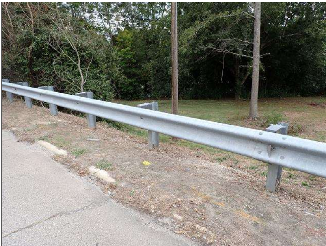
NORTHWEST APPROACH GUARDRAIL POST SPACING AT MID LENGTH, SOUTHWEST AND SOUTHEAST SIMILAR
