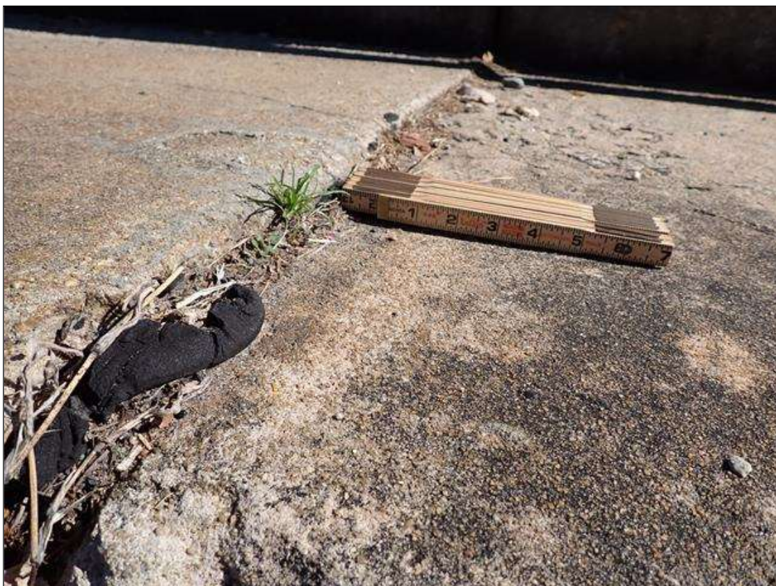
SAG ALONG RIGHT SIDE OF SPAN 3 DECK AND RAIL ABOVE BEAM 7 WITH VERTICAL DEFLECTION OF DECK AND SIEWALK AT BENTS 2 AND 3
