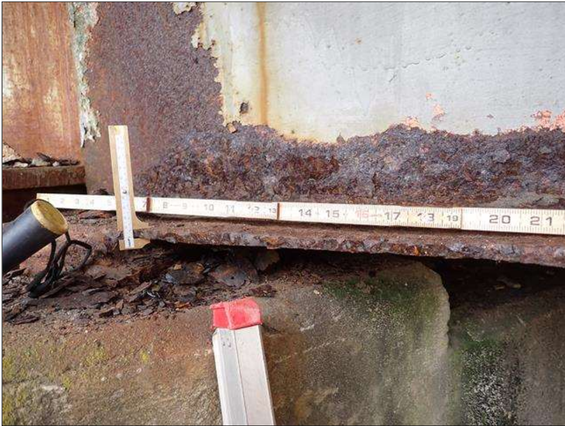
Span 4 Beam 7: PAR: CORROSION ALONG BOTH FACES OF WEB AND BOTTOM FLANGE UP TO 36 INCH LONG X 19 INCH HIGH DOWN TO 3/8 INCH RESIDUAL WEB AND 36 INCH LONG X 10 INCH WIDE DOWN TO 3/8 INCH RESIDUAL BOTTOM FLANGE EXTENDING FROM BENT 3
