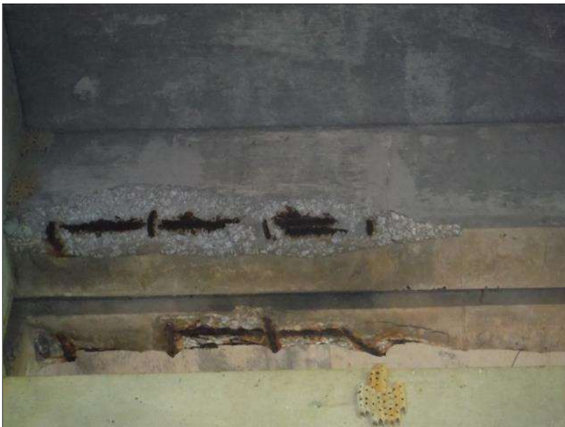
Span 3 Beam 2: (PAR) 3ft x 8in x 2in deep spall with exposed rebar in end diaphragm at bent 2
