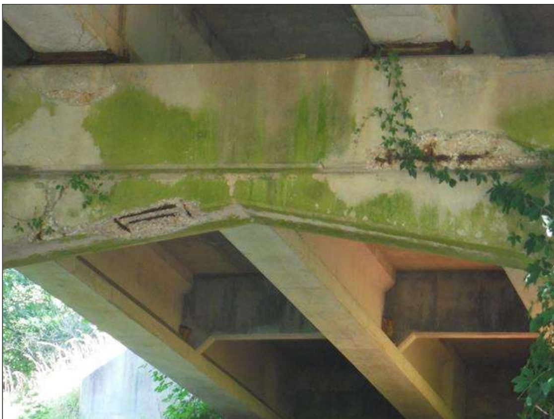
Bent 2 Cap 1: cap south face and bottom between piles 1 and 2. Has a crack/spall and delaminated area with rebar exposed. Area is: from bottom edge up 18", from bottom edge back 21" x 60" long x 2" deep.
