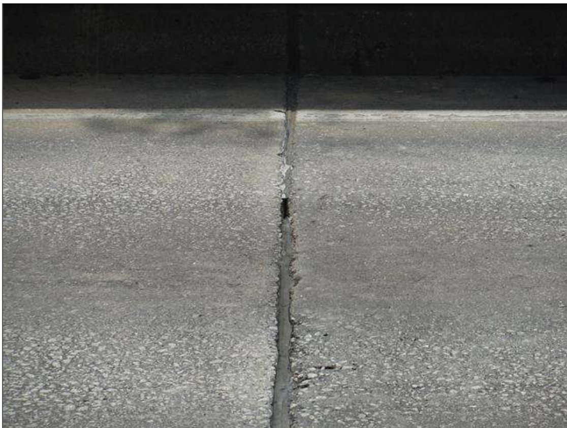
Expansion Joint : over bent 2 has loss of seal adhesion due to cracking along edge in left lane.
