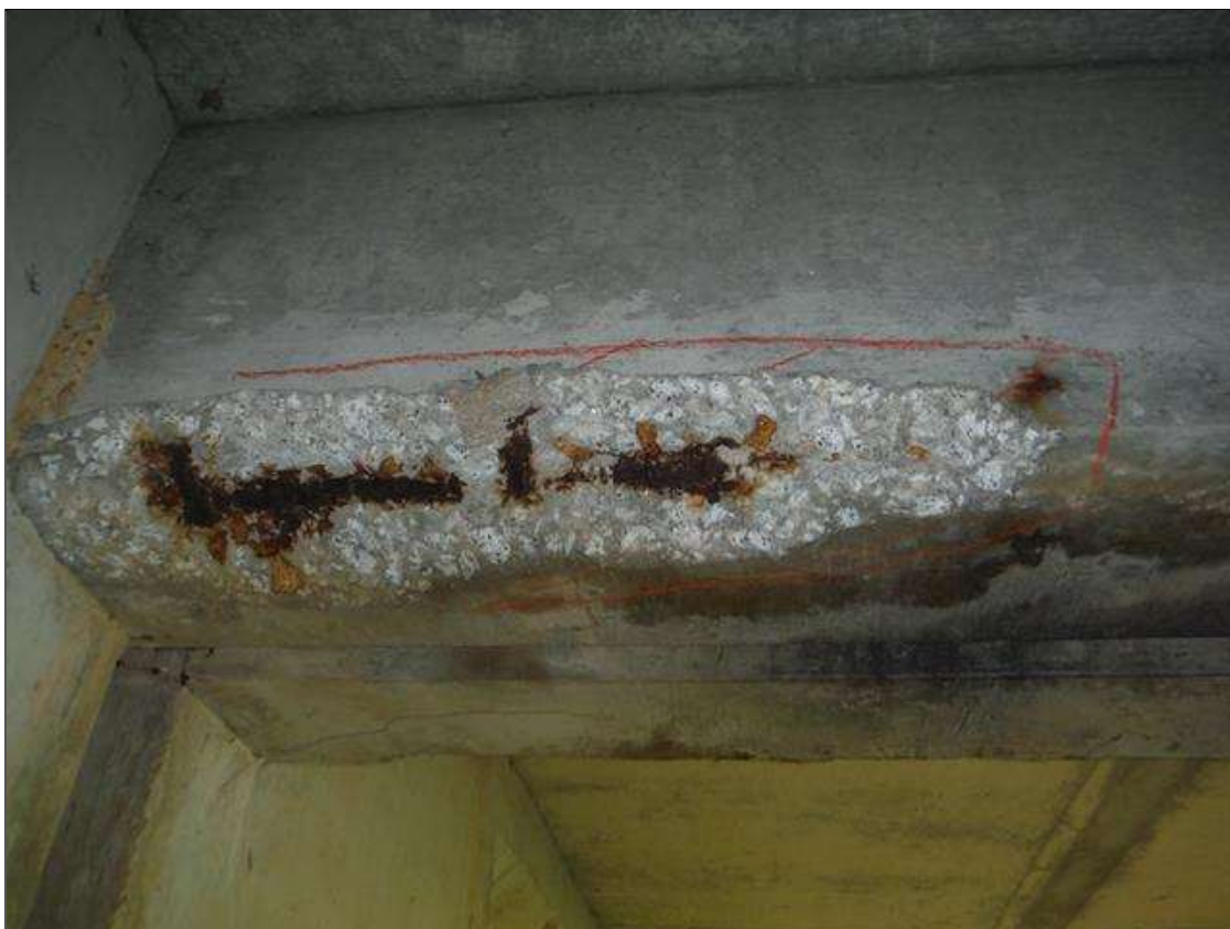
Span 3 Beam 1: (PAR) 2ft x 8in x 2in deep spall with exposed rebar in end diaphragm at bent 2
