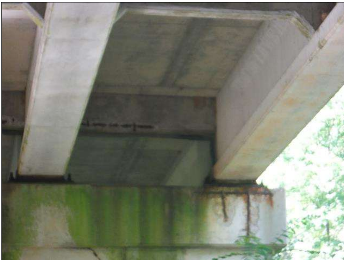
Span 2 Beam 1: (PAR) 3ft x 8in x 2in deep spall with exposed rebar in end diaphragm at bent 1
