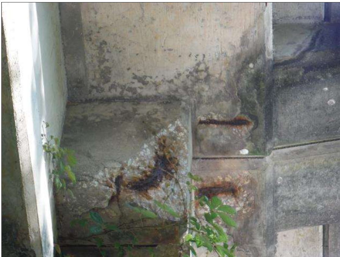
Span 1 Beam 4: (PAR) 2ft x 8in x 2in deep spall with exposed rebar in end diaphragm at bent 1.
