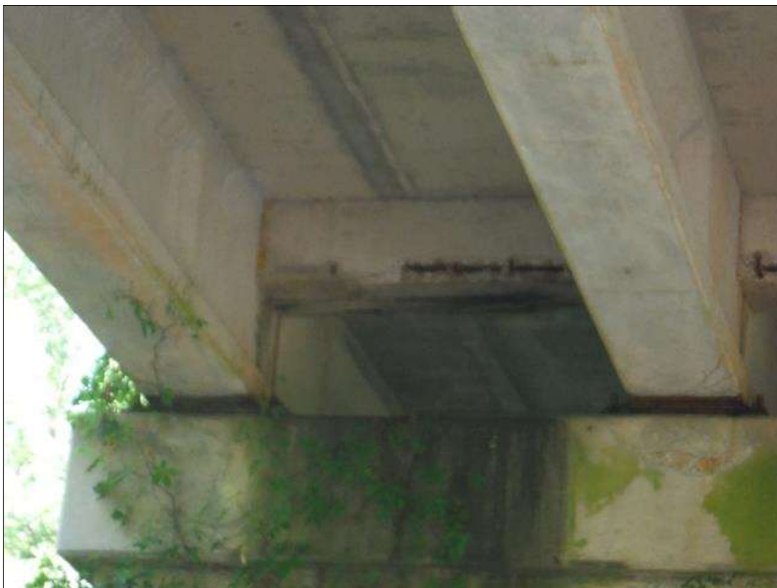
Span 2 Beam 1: (PAR) 4ft x 8in x 2in deep spall with exposed rebar in end diaphragm at bent 2
