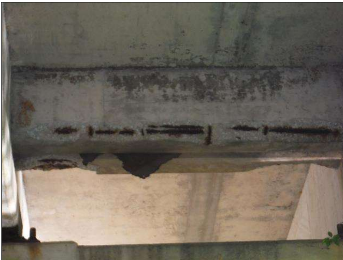
Span 1 Beam 3: (PAR) 4ft x 8in x 2in deep spall with exposed rebar in end diaphragm at bent 1.
