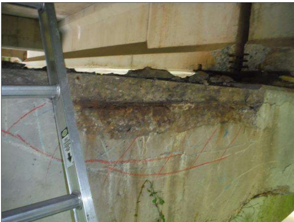
Bent 2 Cap 1: (PAR) cap top, north face in bay 3. Has a crack/spall and delaminated area with rebar exposed. Area is: from top edge down 16", from edge back 12" x 7' x 6" deep.
