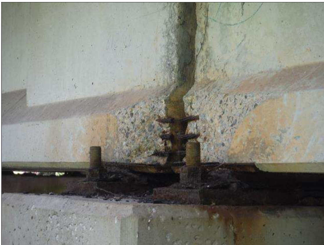
Span 2 Beam 1: (PAR) left bottom flange over bent 1. Has a crack/spall and delaminated with 3 cables exposed. Area is: from bottom edge up 8" x 11" x 2" deep with some section loss to strands.
