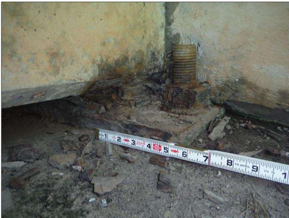
Span 1 Beam 1 Near Bearing: has scattered rust and flaking, anchor nut has 50 percent section loss.
