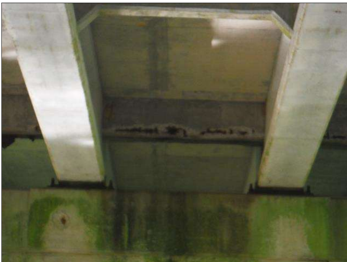
Span 2 Beam 2: (PAR) 4ft x 8in x 2in deep spall with exposed rebar in end diaphragm
