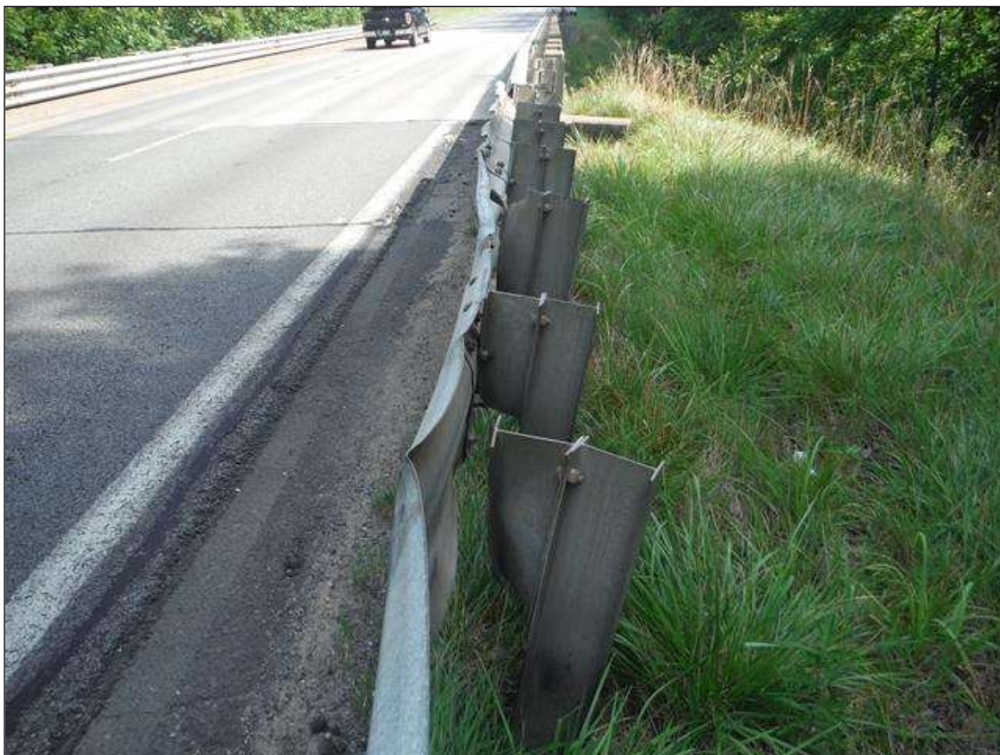
(PAR) 20ft impact damage to far left guardrail at end bent 2
