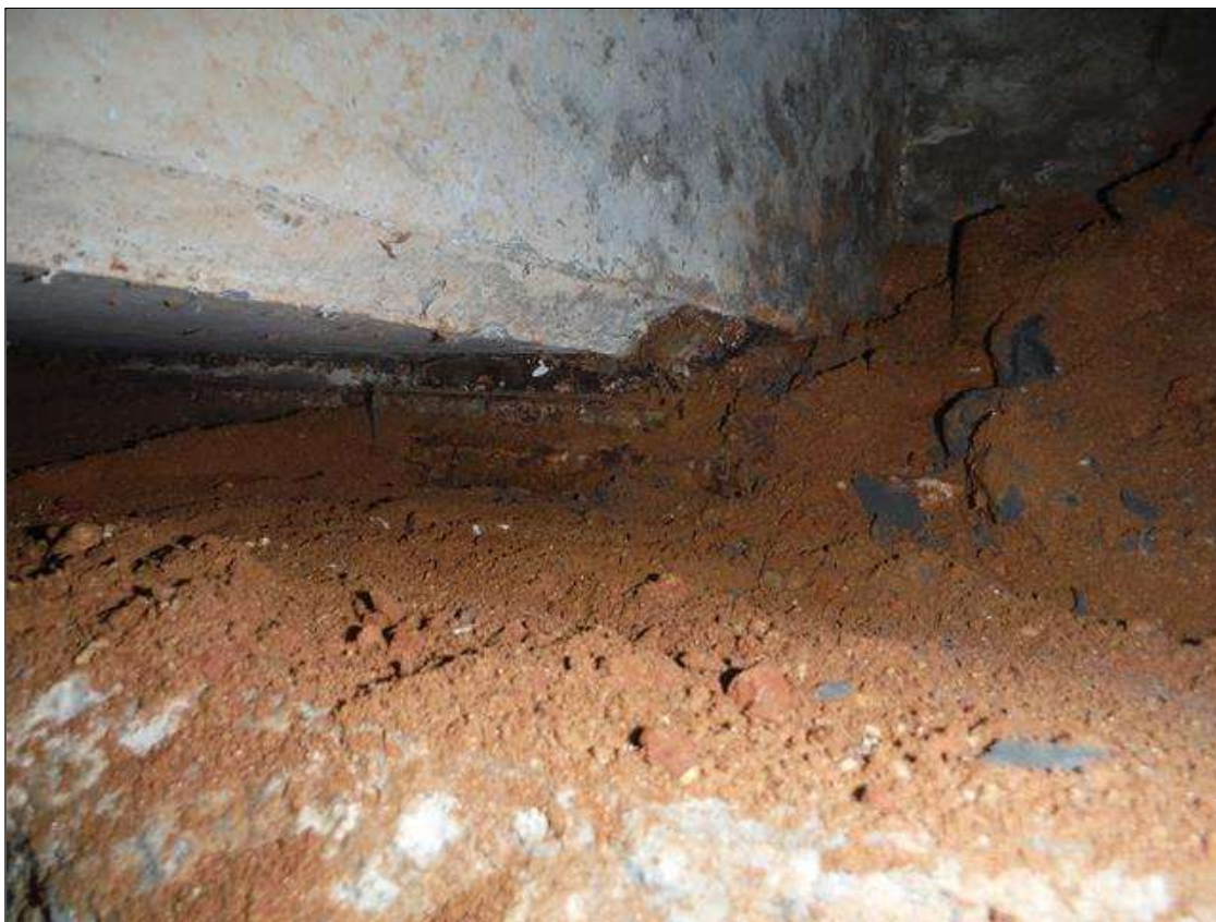
Span 1 Beam 2 Near Bearing: surface corrosion and covered in dirt.
