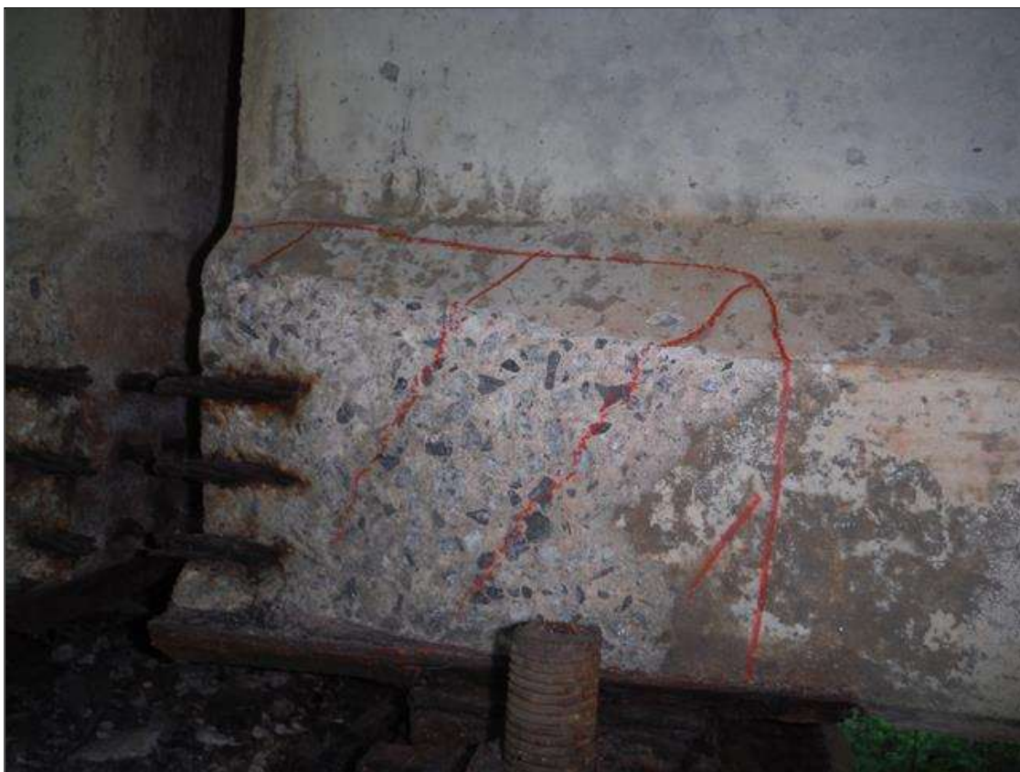
Span 3 Beam 4: (PAR) right bottom flange over bent 2. Has a spalled area with 3 cables exposed. Area is: 8" x 15" x 2" deep with some section loss to strands.
