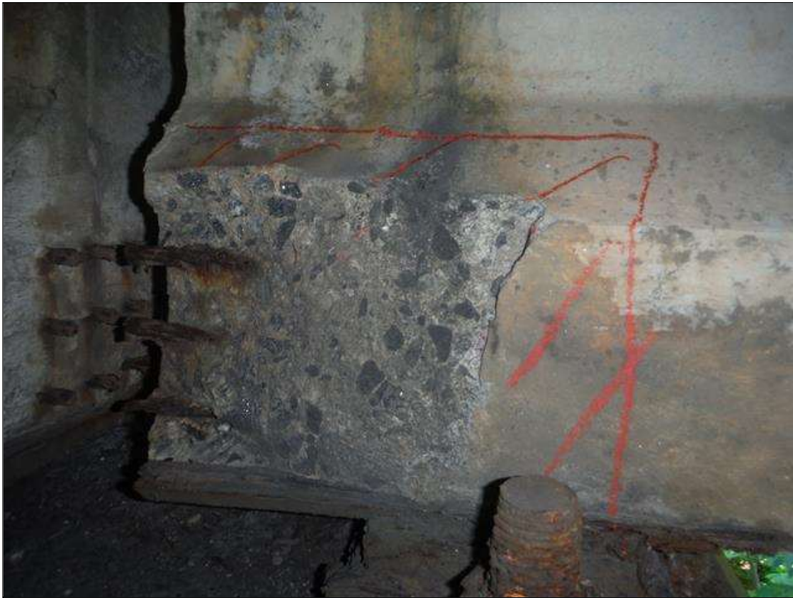
Span 3 Beam 1: (PAR) right bottom flange over bent 2. Has a crack/spall and delaminated area with 3 cables exposed. Area is: from bottom up 7" x 9" x 1 1/2" deep with some section loss to strands.
