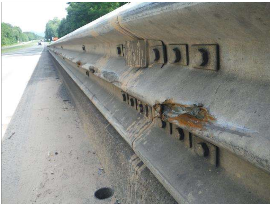
Span 2 Left Bridge Rail: has torn areas due to impact damage.
