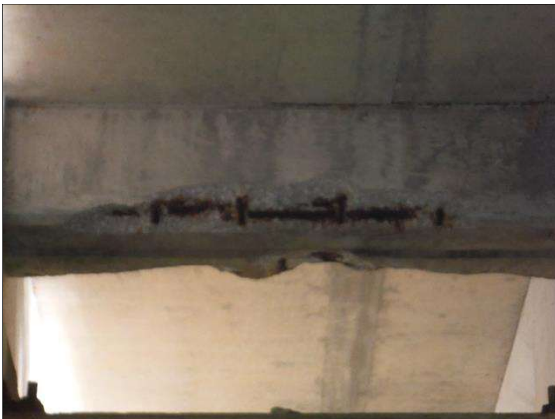
Span 1 Beam 2: (PAR) 3ft x 8in x 2in deep spall with exposed rebar in end diaphragm at bent 1.
