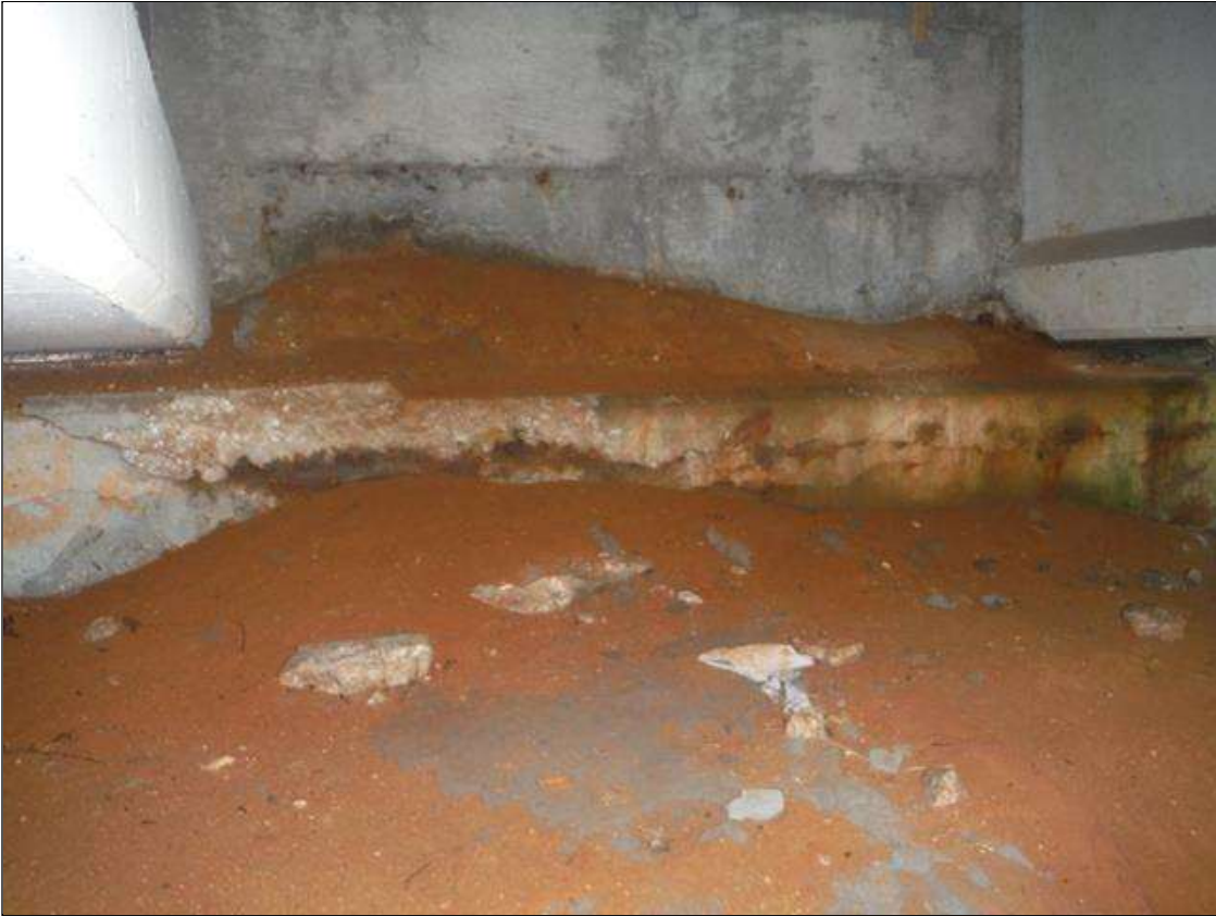
End Bent 1 Cap 1: north face bay 1, has a crack/spall and delaminated area with rebar exposed. Area is: from top edge down 9in x 8ft x 2in deep.
