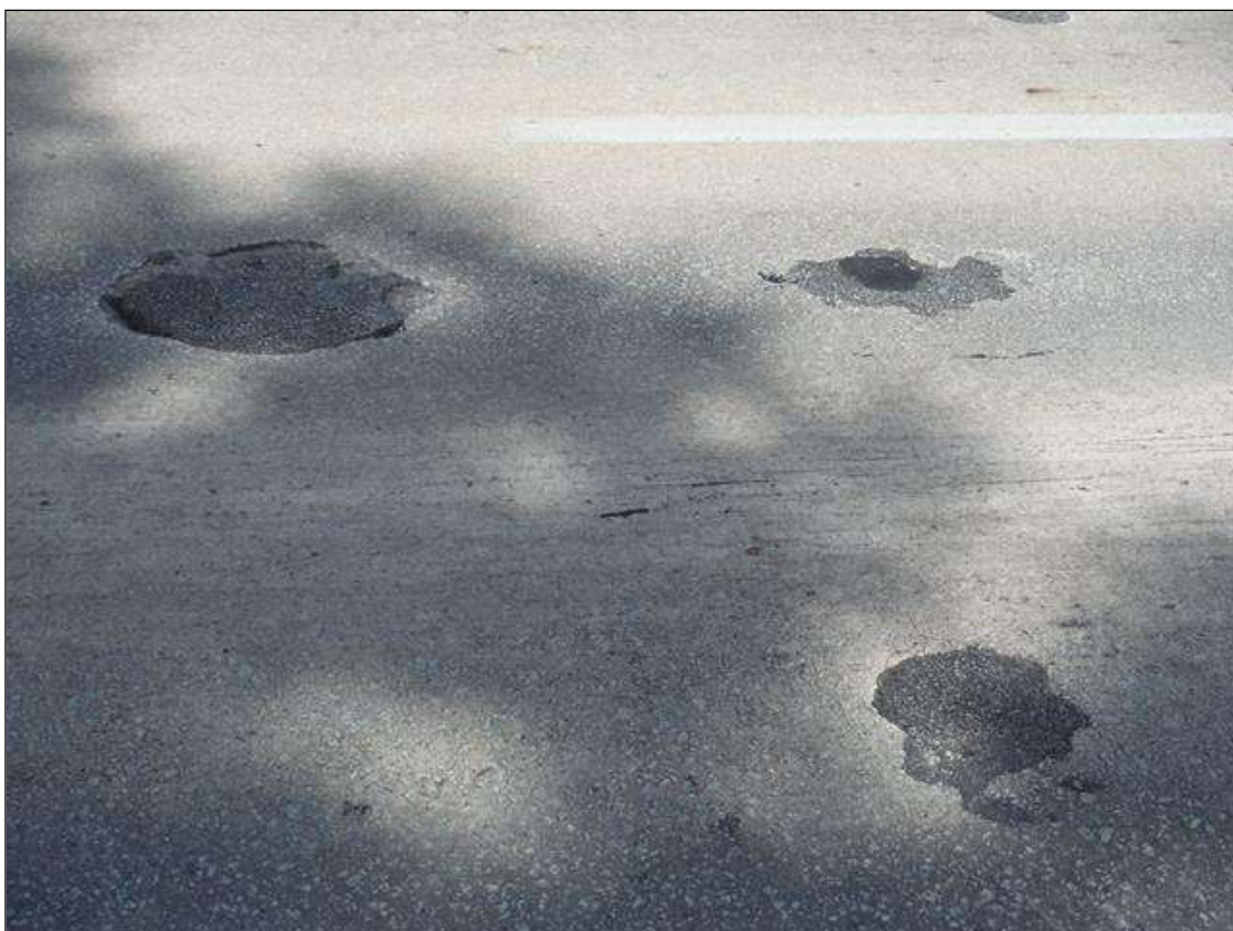
Span 1 Deck: top of deck left lane has scattered patches. patches are from: 10" x 10" up to 20" x 20".
