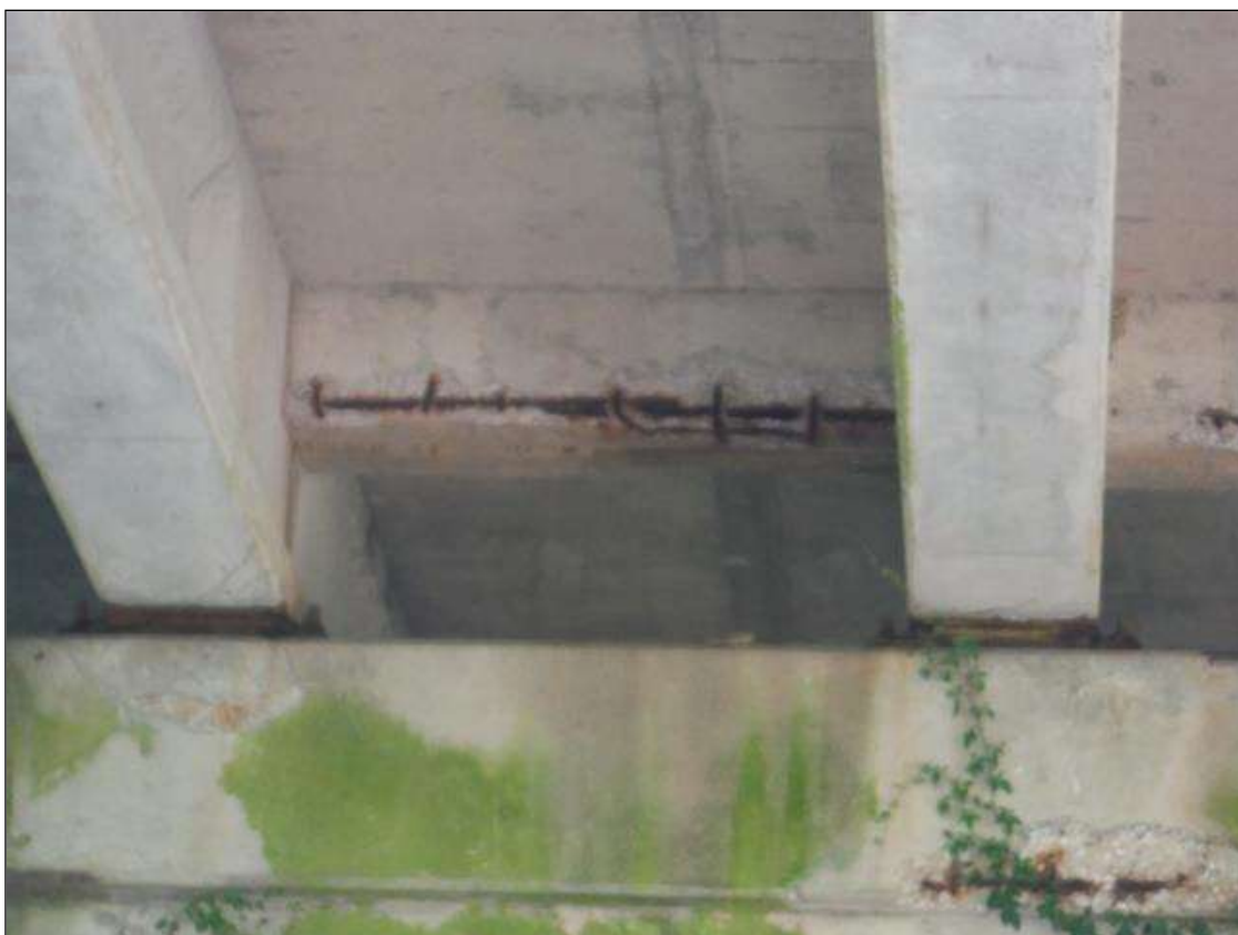
Span 2 Beam 2: (PAR) 4ft x 8in x 2in deep spall with exposed rebar in end diaphragm at bent 2
