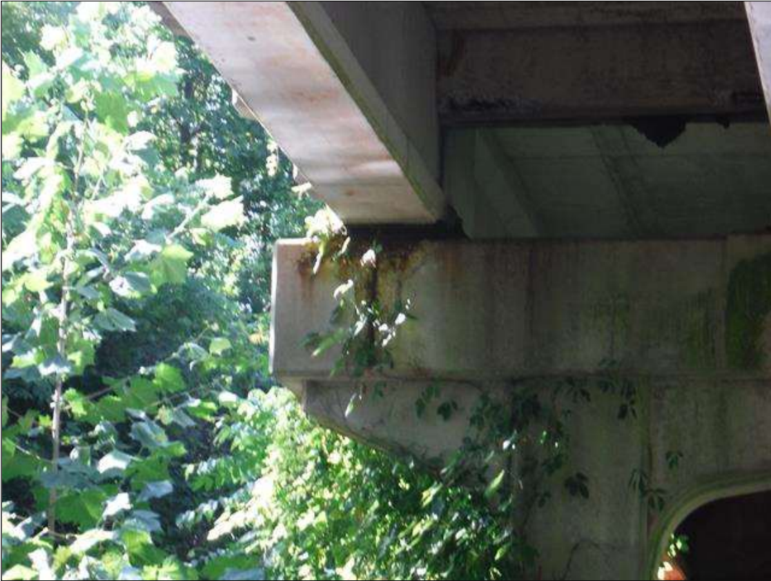
Bent 1 Cap 1: (PAR) cap north face at beam 4. Has a crack/spall and delaminated area with rebar exposed. Area is: from top edge back 2", from top edge down 30" x 36" x 2" deep. With heavy rust and flaking on rebar.
