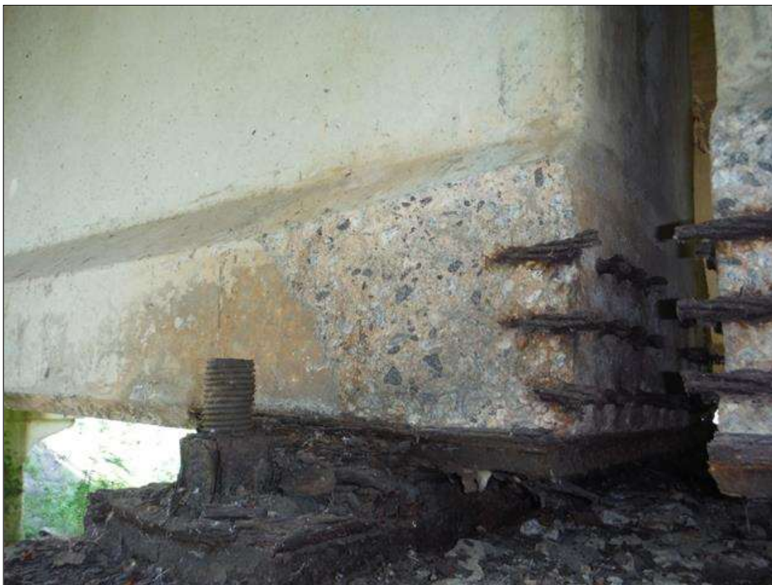
Span 2 Beam 4: (PAR) right bottom flange over bent 2. Has a crack/spall and delaminated area with 3 cables exposed. Area is: 8" x 13" x 1 1/2" deep with some section loss on strands.
