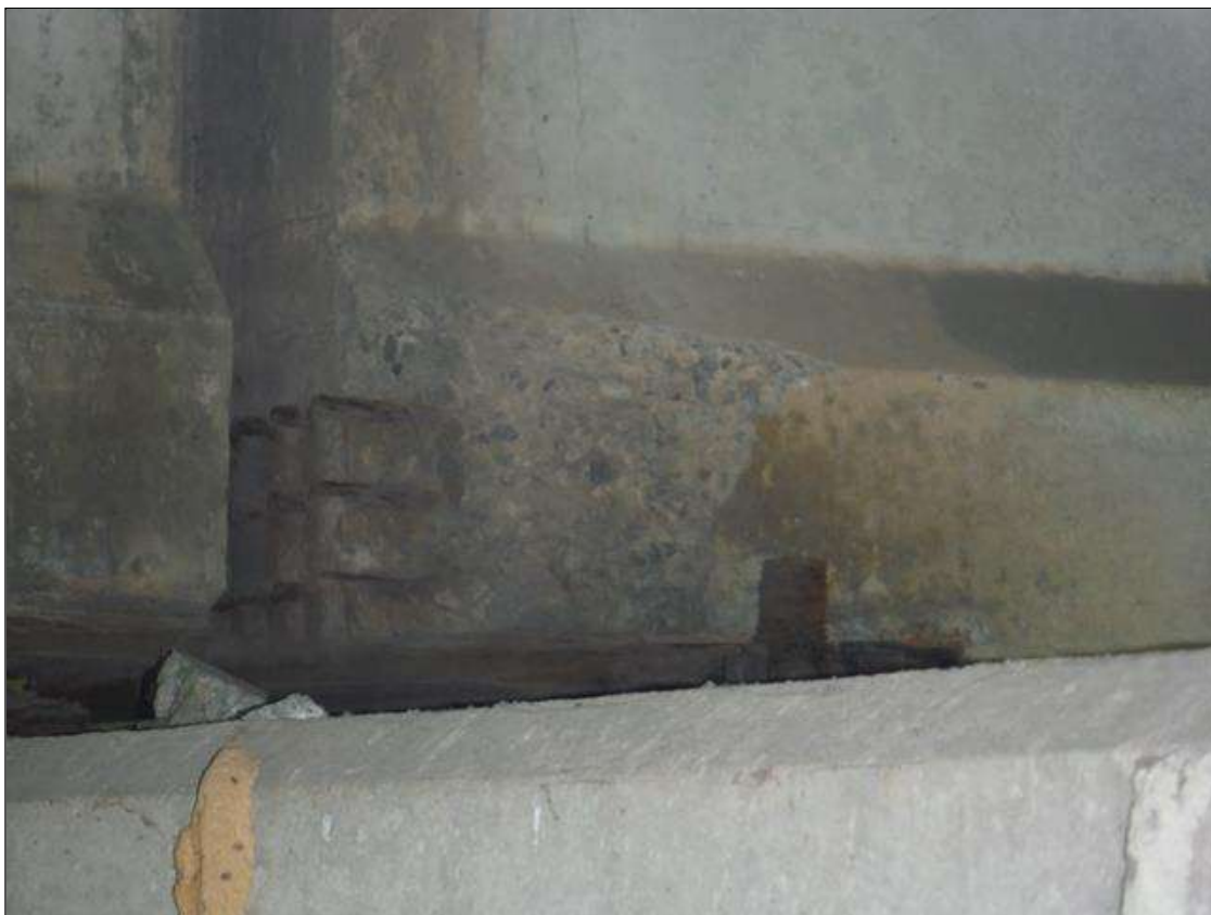
Span 2 Beam 3: (PAR) left bottom flange over bent 2. Has a crack/spall and delaminated area with cables exposed. Area is: from bottom up 8" x 10" x 2" deep with some section loss to strands.
