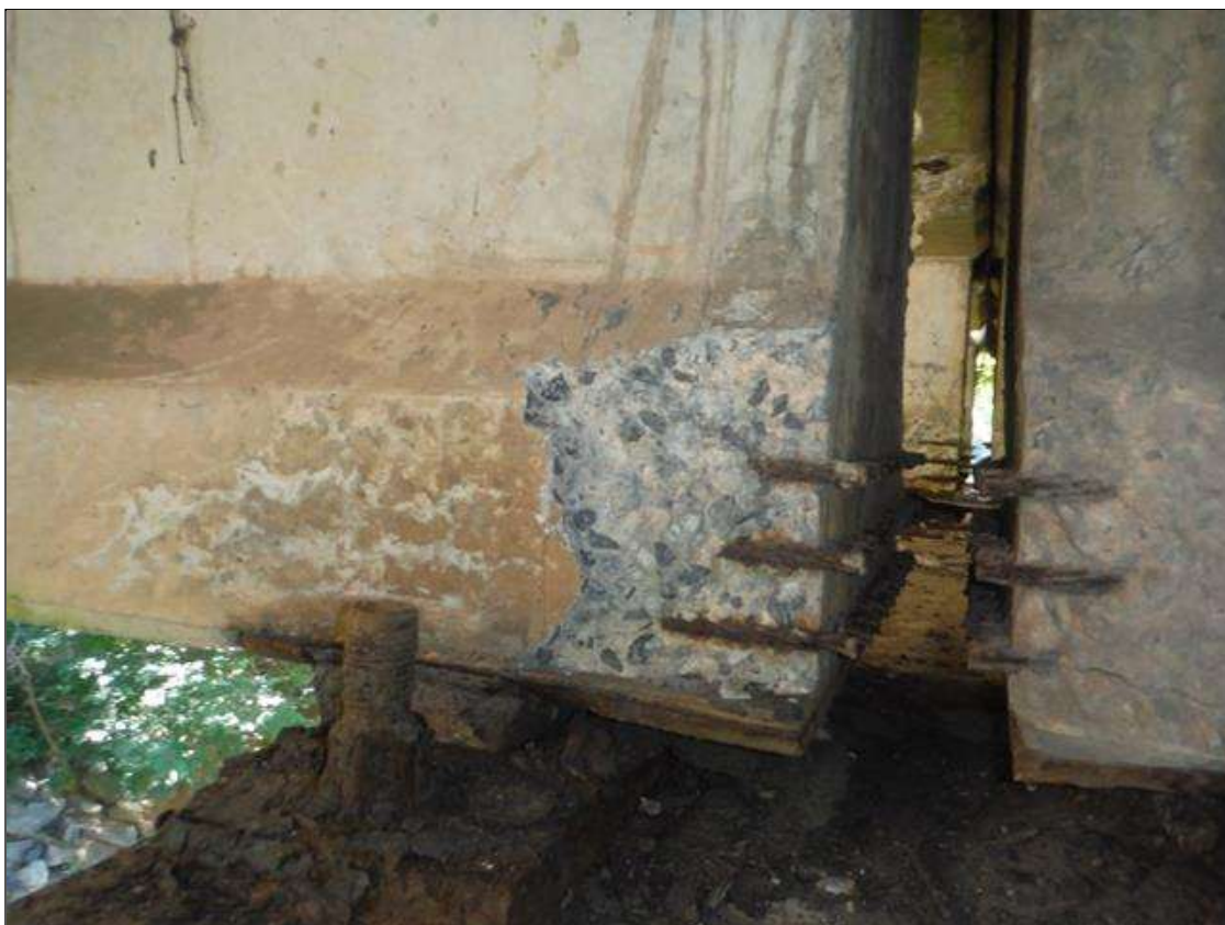
Span 2 Beam 2: (PAR) left bottom flange over bent 1. Has a crack/spall and delaminated area with 3 cables exposed. Area is: from bottom up 8" x 8" x 2" deep with minor section loss to strands.
