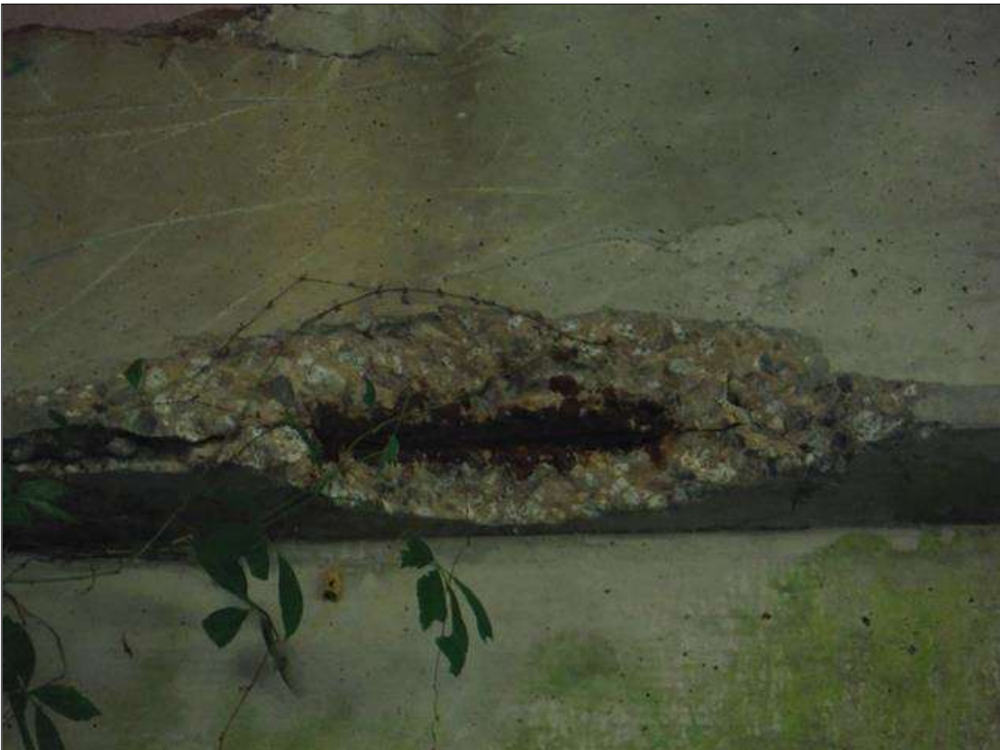
Bent 2 Cap 1: (PAR) cap bottom and north face at beam 3. Has a crack/spall and delaminated area with rebar exposed. Area is: from bottom edge up 12", from bottom edge back 7" x 43" long x 5" deep.
