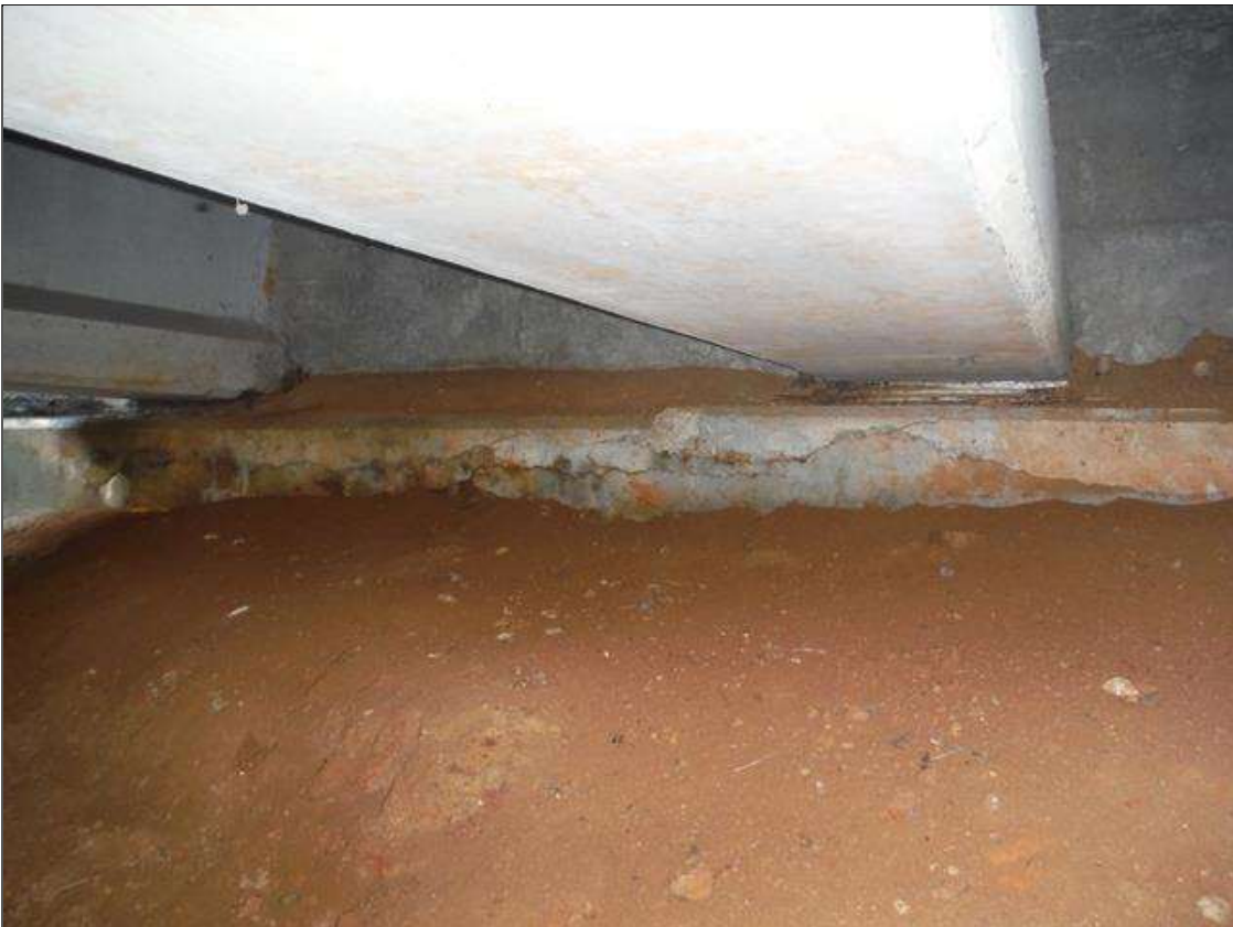
End Bent 1 Cap 1: north face has a crack/spall and delaminated area with efflorescence and rust stains visible. Area begins left of beam 3 and extends to right of beam 4. Area is: from top edge down 9in x 11ft long x 1in deep.
