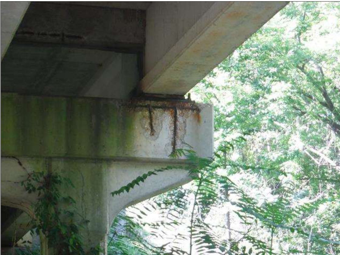
Bent 1 Cap 1: (PAR) cap north face under beam 1. Has a crack/spall and delaminated area with rebar exposed. Area is: from top edge back 3", from top edge down 29" x 54" x 1 1/2" deep with some heavy rust and flaking to rebar.
