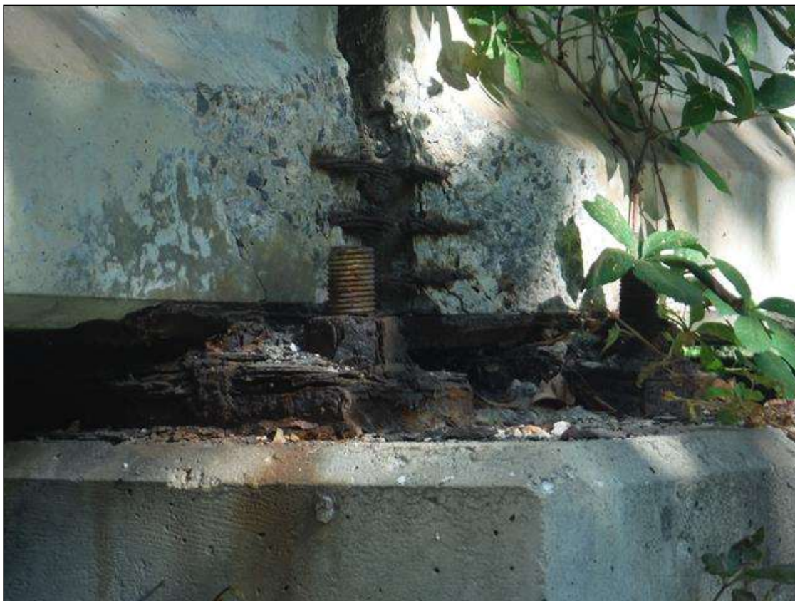
Span 1 Beam 4: (PAR) right bottom flange over bent 1. Has a crack/spall and delaminated area with 3 cables exposed. Area is: from bottom up 10" x 17" x 2" deep with minor section loss to strands.
