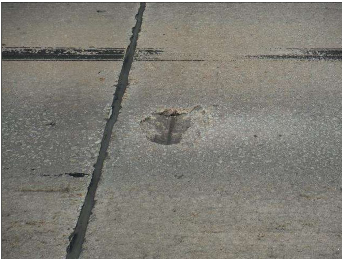
Span 1 Deck: (PAR) 1ft diameter by 1in spall with exposed rebar in left lane at bent 1 joint
