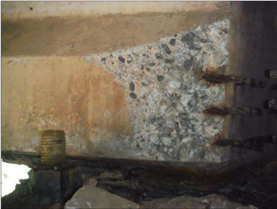
Span 2 Beam 3: (PAR) right bottom flange over bent 2. Has a crack/spall and delaminated area with 3 cables exposed. Area is: from bottom edge up 8" x 10" x 2" deep. Strands appear to have some section loss.
