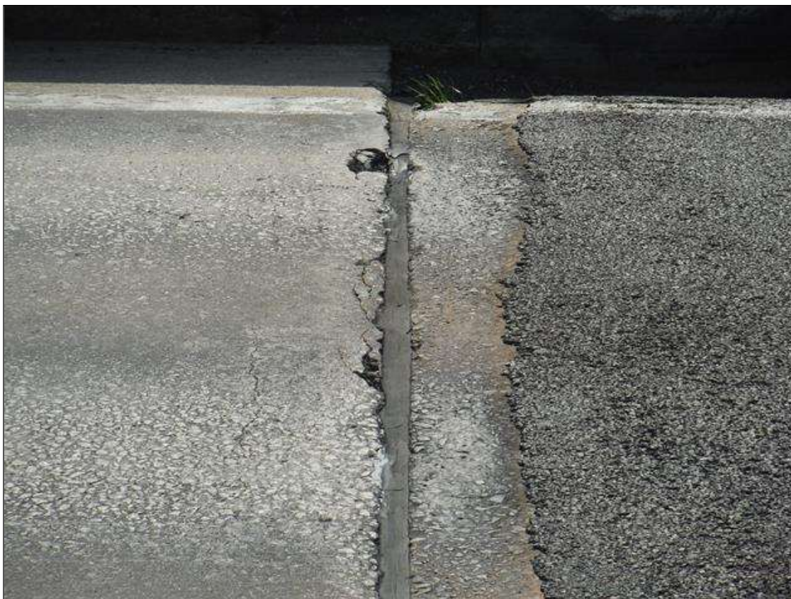
Span 3 Deck: 3ft x 6in x 1in deep cracking and spall in left lane at end bent 2 joint
