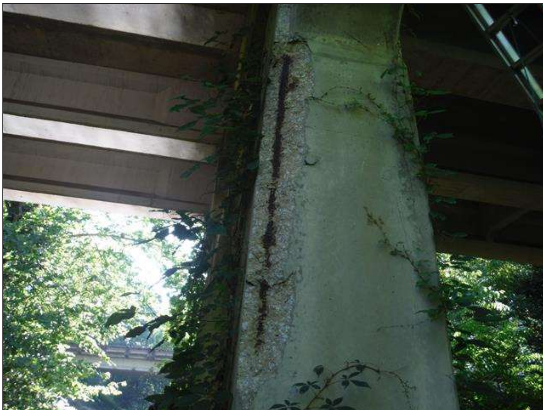
Bent 1 Pile 1: (PAR) northwest corner has a crack/spall and delaminated area. Located 16" below bottom of cap. Area on north face is: 6", area on west face is: 9" x 92" long.
