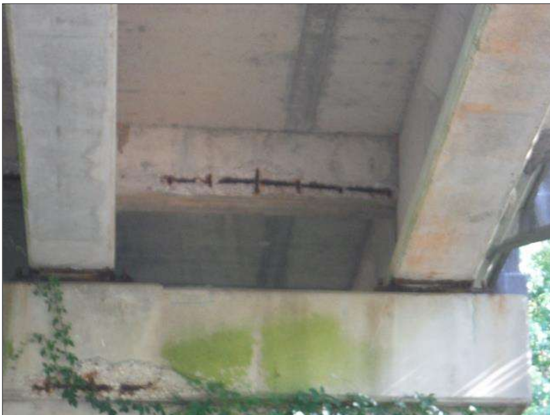
Span 2 Beam 3: (PAR) 4ft x 8in x 2in deep spall with exposed rebar in end diaphragm at bent 2
