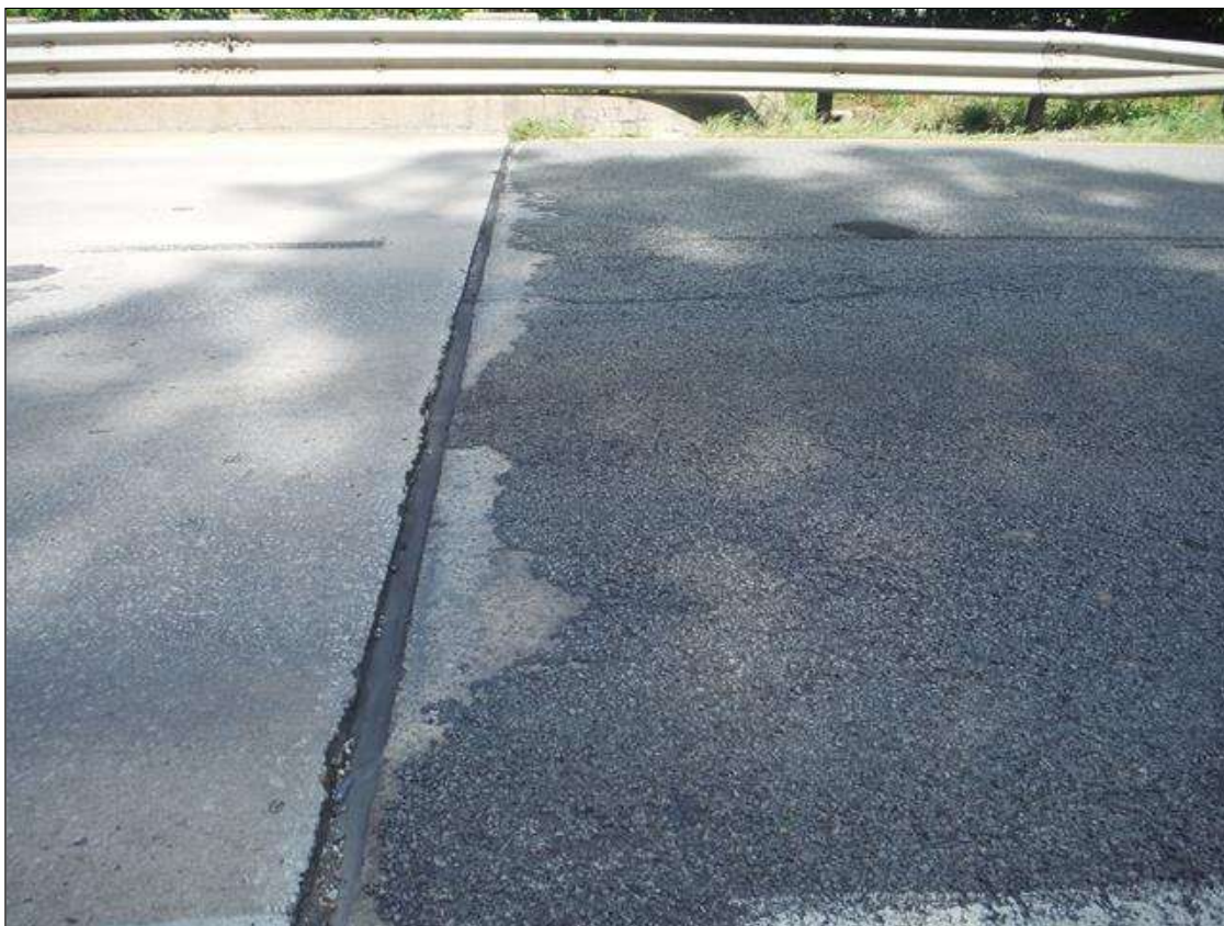
Approach 1: full width by 2ft of missing asphalt wearing surface at joint
