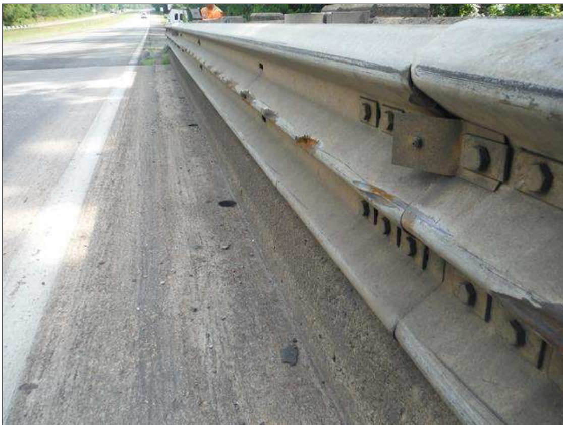
Span 1 Left Bridge Rail: has torn areas due to impact damage.
