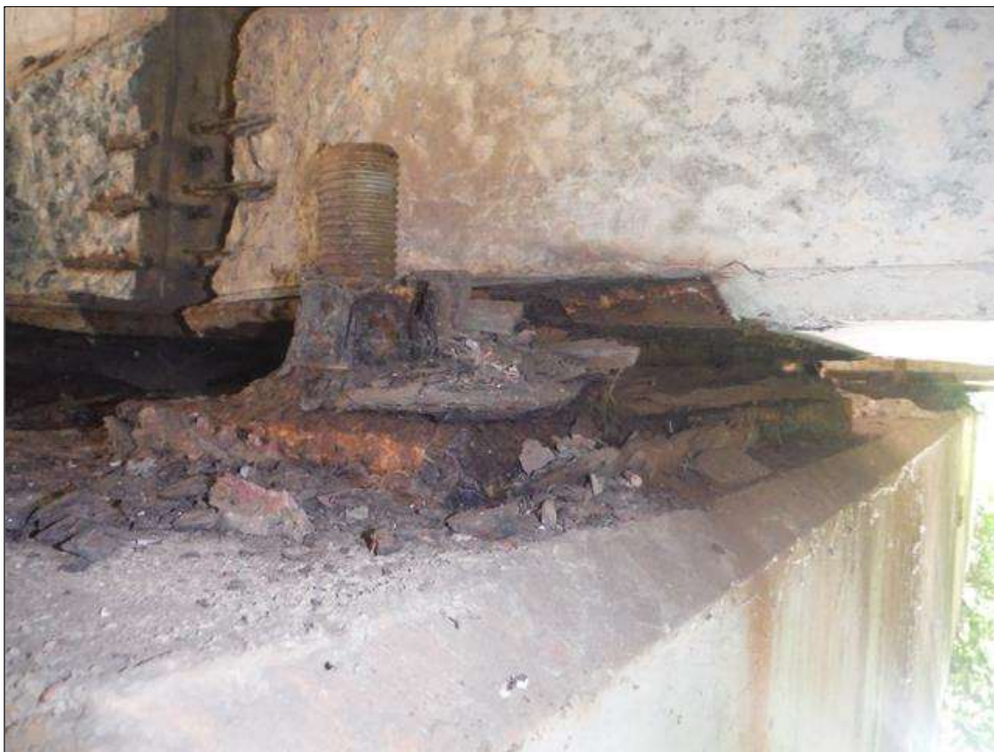
Span 1 Beam 2 Far Bearing: heavy corrosion and scaling with up to 1/4in section loss, typical all bearing at bent 1 and bent 2.
