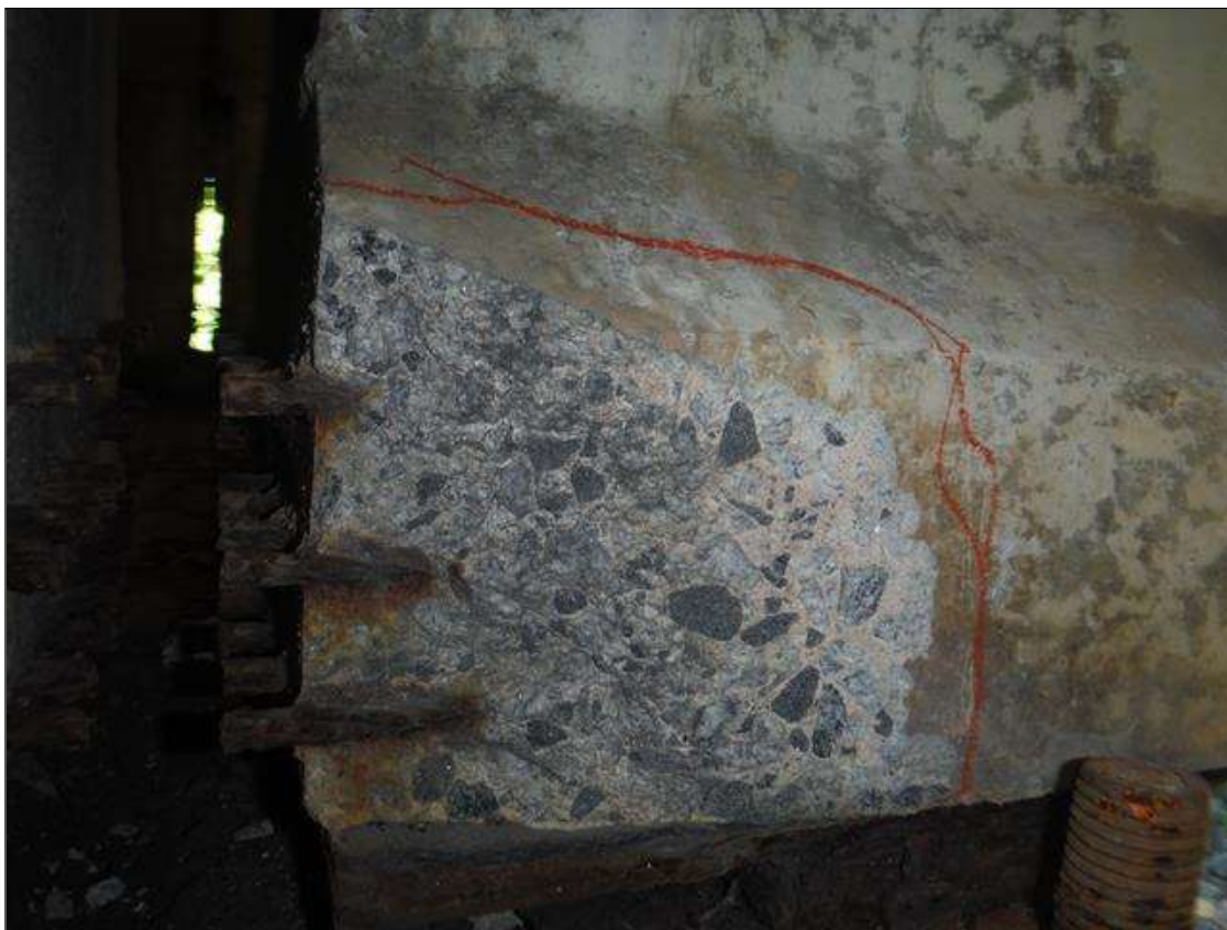
Span 2 Beam 3: (PAR) right bottom flange over bent 1. Has a crack/spall and delaminated area with 3 cables exposed. Area is: from bottom up 8" x 8" x 2" deep with minor section loss to strands.
