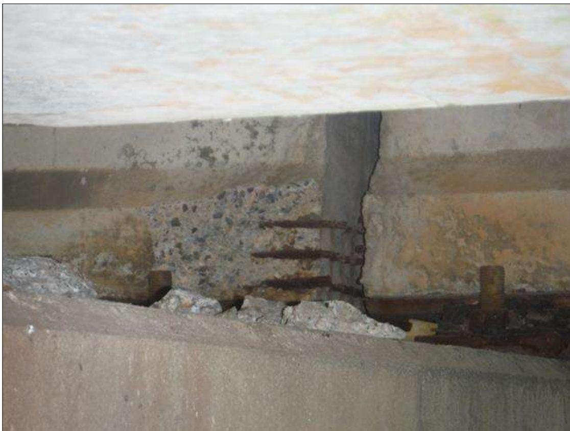
Span 2 Beam 3: (PAR) left bottom flange over bent 1. Has a crack/spall and delaminated area with 3 cables exposed. Area is: from bottom up 8" x 12" x 2" deep with minor section loss to strands.
