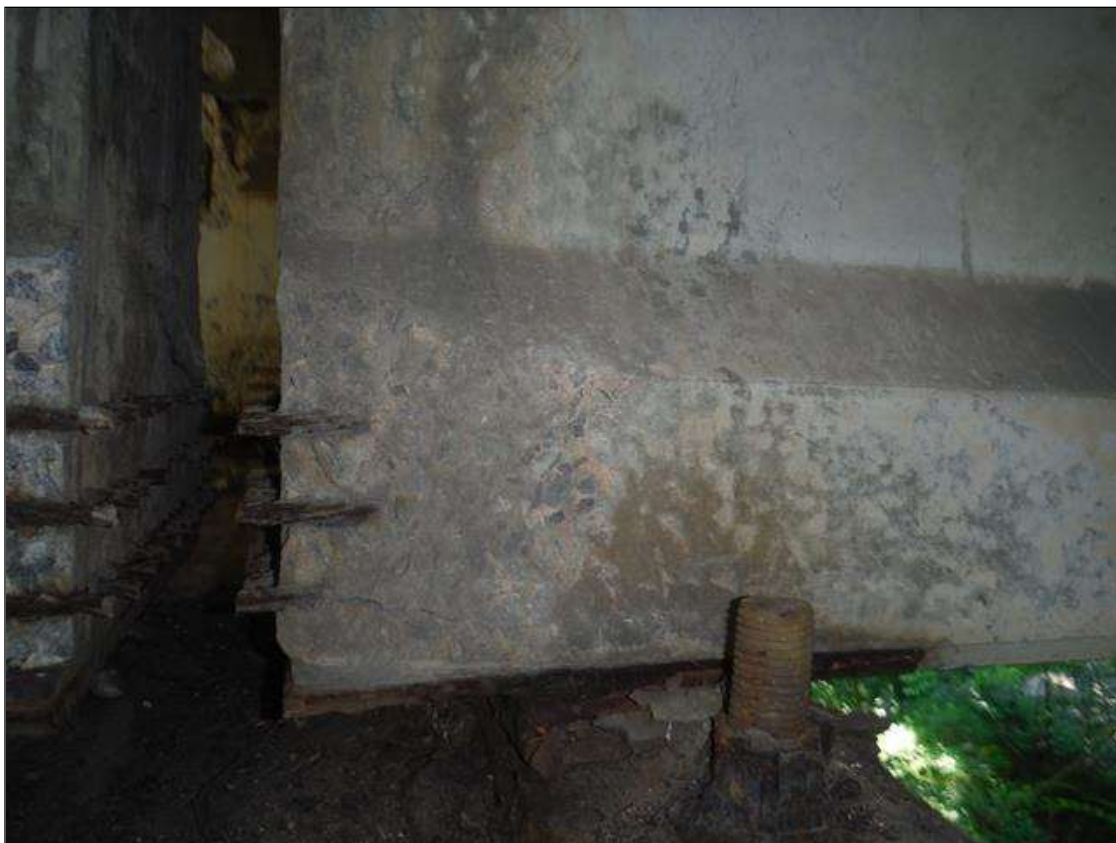
Span 1 Beam 2: (PAR) left bottom flange at bent 1. Has a crack/spall and delaminated area with 3 cables exposed. Area is: from bottom up 9" x 10" x 2" deep with minor section loss to strands.
