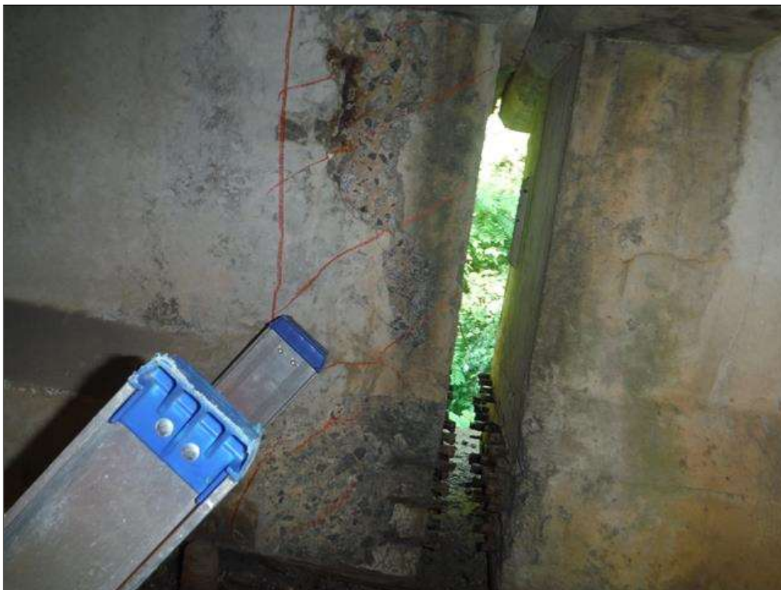
Span 1 Beam 1: (PAR) right bottom flange over bent 1. Has a crack/spall and delaminated area with 3 cables exposed. Area is: from bottom up 8" x 11" x 2" deep with minor section loss to strands.
