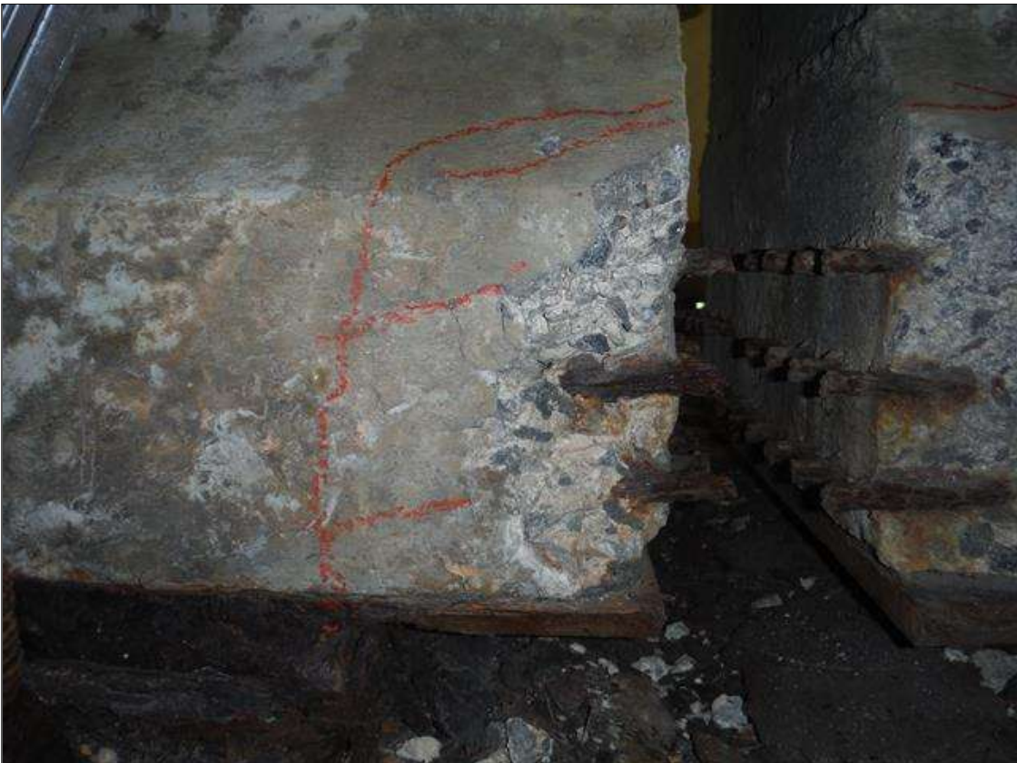
Span 1 Beam 3: (PAR) right bottom flange over bent 1. Has a crack/spall and delaminated area with 2 cables exposed. Area is: from bottom up 8" x 8" x 2" deep with minor section loss to strands.
