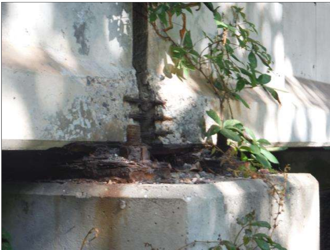
Span 2 Beam 4: (PAR) right bottom over bent 1. Has a crack/spall and delaminated area with 3 cables exposed. Area is: from bottom up 10" x 14" x 2" deep with minor section loss to strands.
