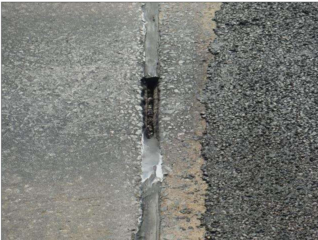
Expansion Joint : over end bent 2 has loss of seal adhesion due to cracking along edge. Material is missing in right lane.
