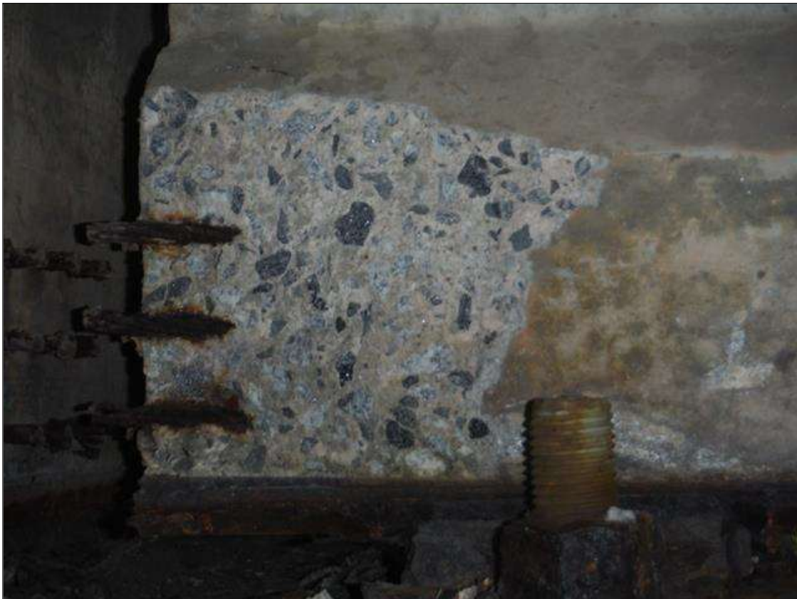
Span 3 Beam 3: (PAR) right bottom flange over bent 2. Has a crack/spall and delaminated area with 3 cables exposed. Area is: from bottom up 8" x 10" x 2" deep. Strands appear to have some section loss.
