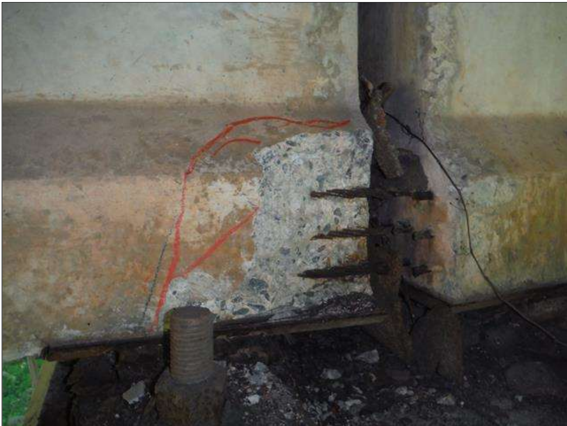
Span 3 Beam 2: (PAR) left bottom flange at bent 2. Has a crack/spall and delaminated area with 3 cables exposed. Area is: from bottom up 8" x 11" x 1 1/2" deep. Strands appear to have some section loss.
