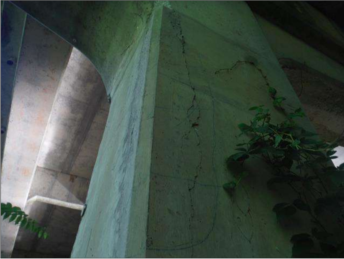
Bent 1 Pile 1: Bent 1 pile 1 southwest corner. Has a crack/spall and delaminated area. Area on west face is: 5", area on south face is: 9" x 60" x 2" deep.
