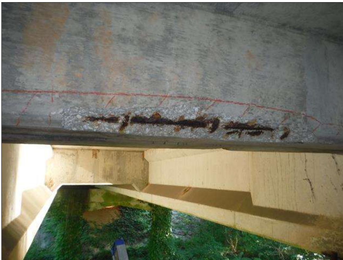
Span 1 Beam 1: (PAR) 4ft x 8in x 2in deep spall with exposed rebar in end diaphragm at bent 1.
