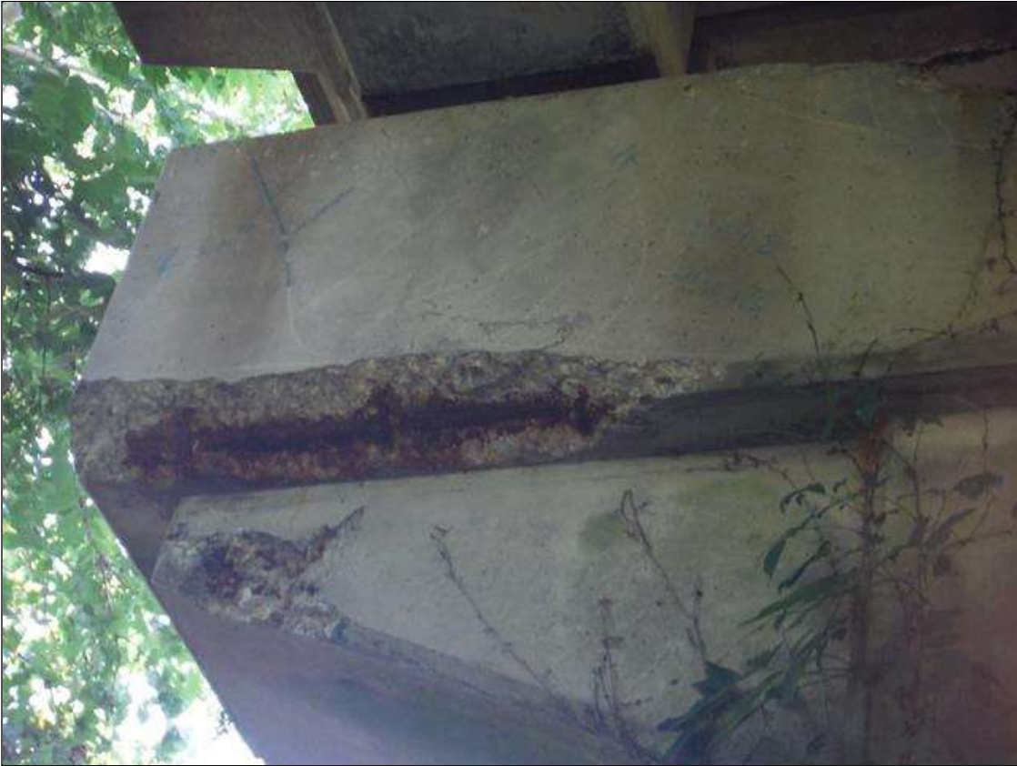
Bent 2 Cap 1: (PAR) cap top, north face and bottom at beam 4. Has a crack/spall and delaminated area with rebar exposed. Area is: from top down 28", from top edge back 2", from bottom edge back 7" x 48".
