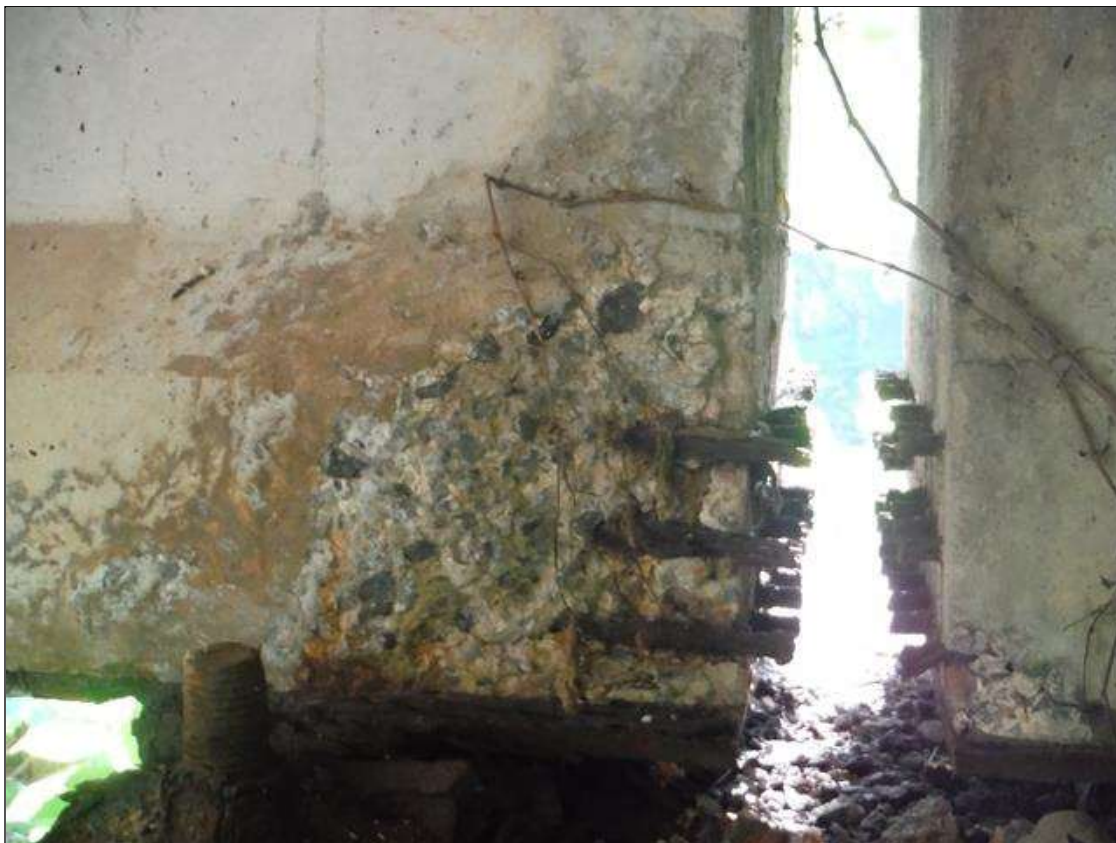
Span 2 Beam 4: (PAR) left bottom flange over bent 1. Has a crack/spall and delaminated area with 3 cables exposed. Area is: from bottom up 9" x 9" x 2" deep with minor section loss to strands.
