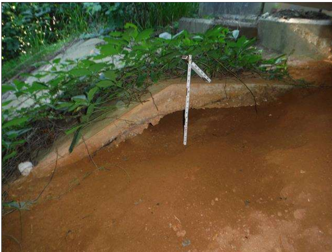
(PAR) near right slope protection is undermined 4ft deep x 3ft x 9in
