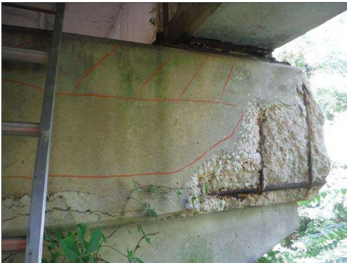
Bent 2 Cap 1: (PAR) cap north face at beam 1. Has a crack/spall and delaminated area with rebar exposed. Area is: from top edge back 2", from bottom edge back 7", from top down 29" x 7' long x 2" deep with heavy rust and flaking on rebar.
