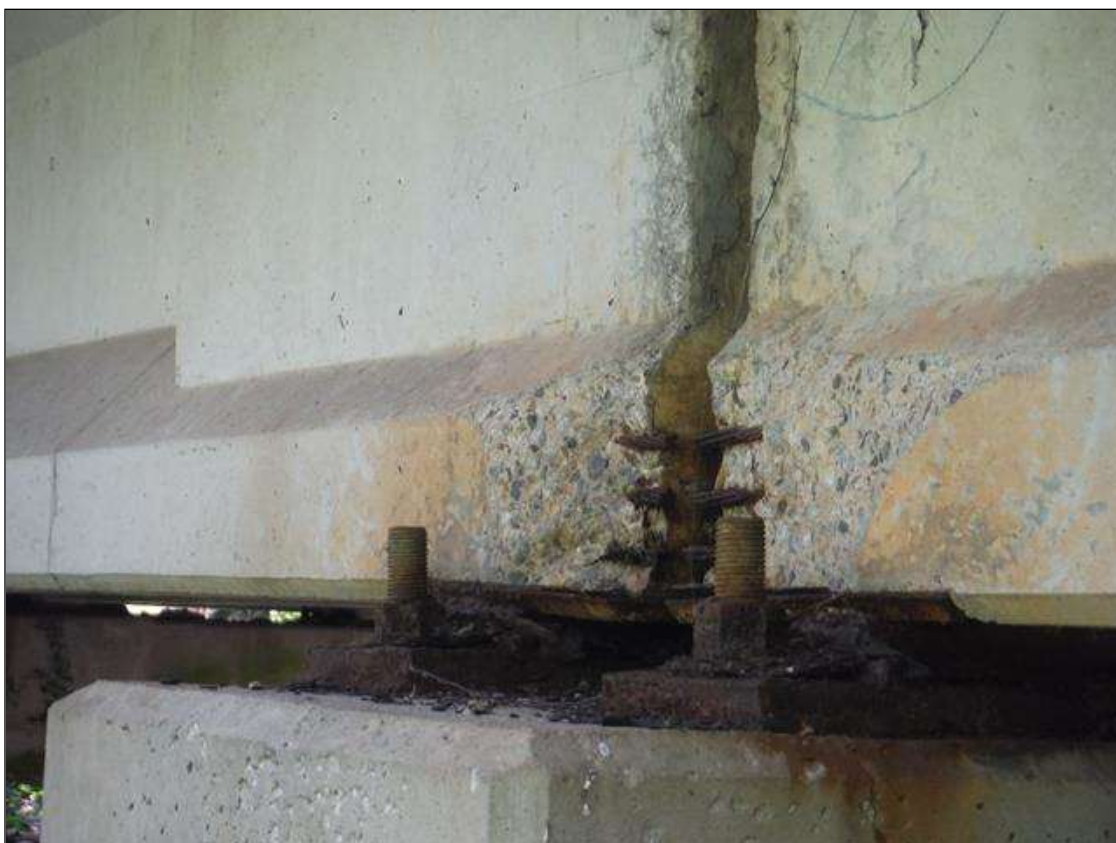
Span 1 Beam 1: (PAR) left bottom flange over bent 1. Has a crack/spall and delaminated area with 3 cables exposed. Area is: from bottom edge up 8" x 21" x 2" deep with minor section loss to strands.
