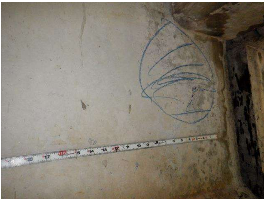
Span 1 Beam 2: East face at far end, delamination [12in diameter]
