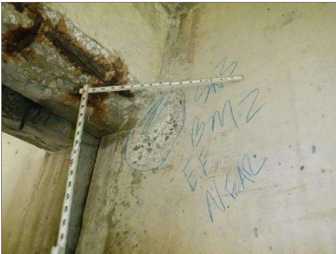
Span 3 Beam 2: East face at near end, spall/delamination [8in x 10in x 3/4in deep]
