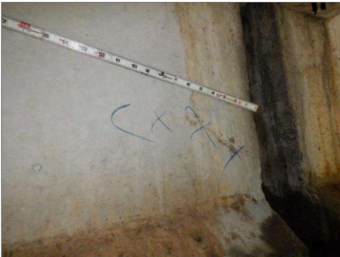
Span 1 Beam 3: East face at far end, diagonal crack [12in x up to 0.004in]
