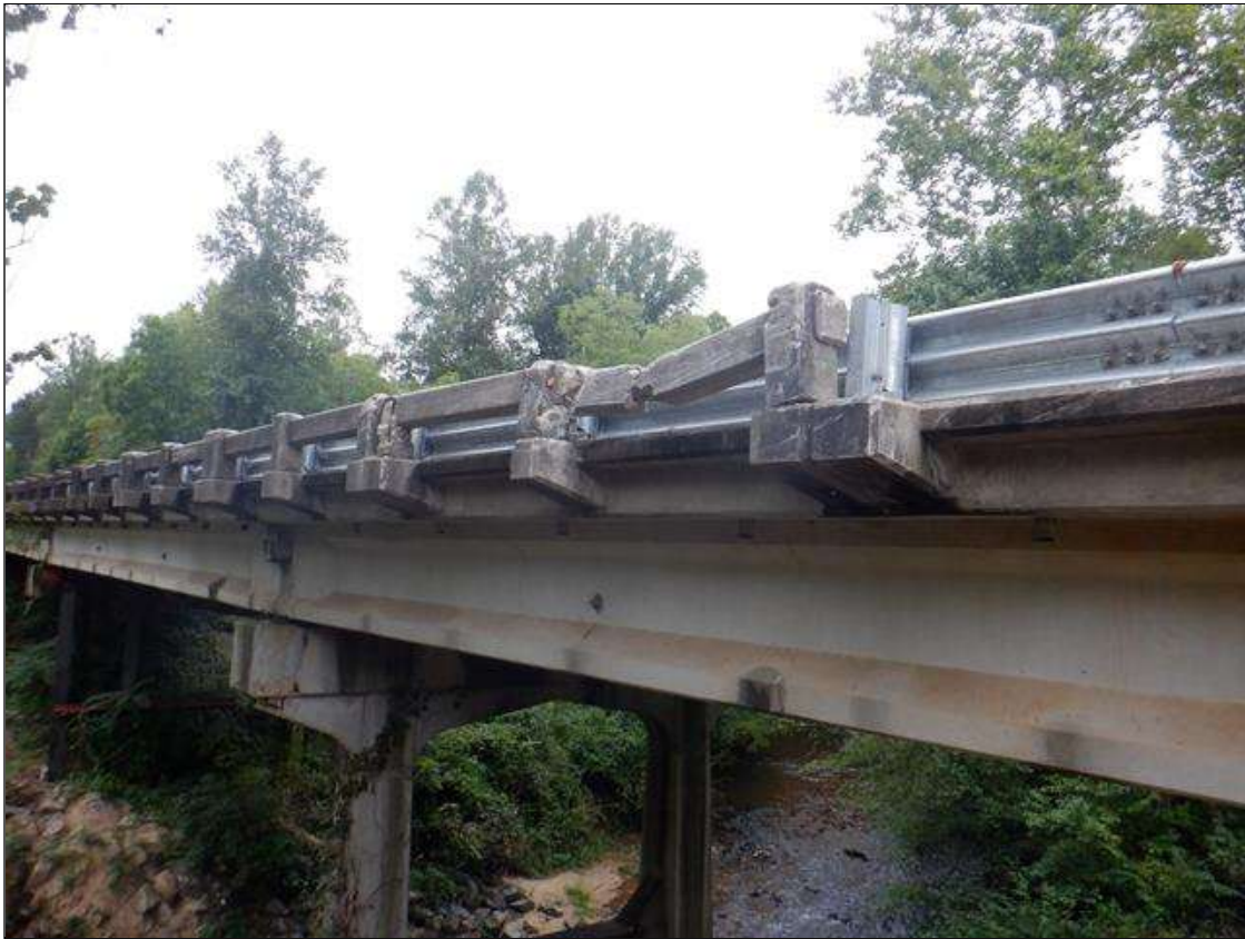
Span 1 Left Bridge Rail: [PAR] at near end, vehicular impact damage [2/3 of length missing], repair crew onsite at time of inspection
