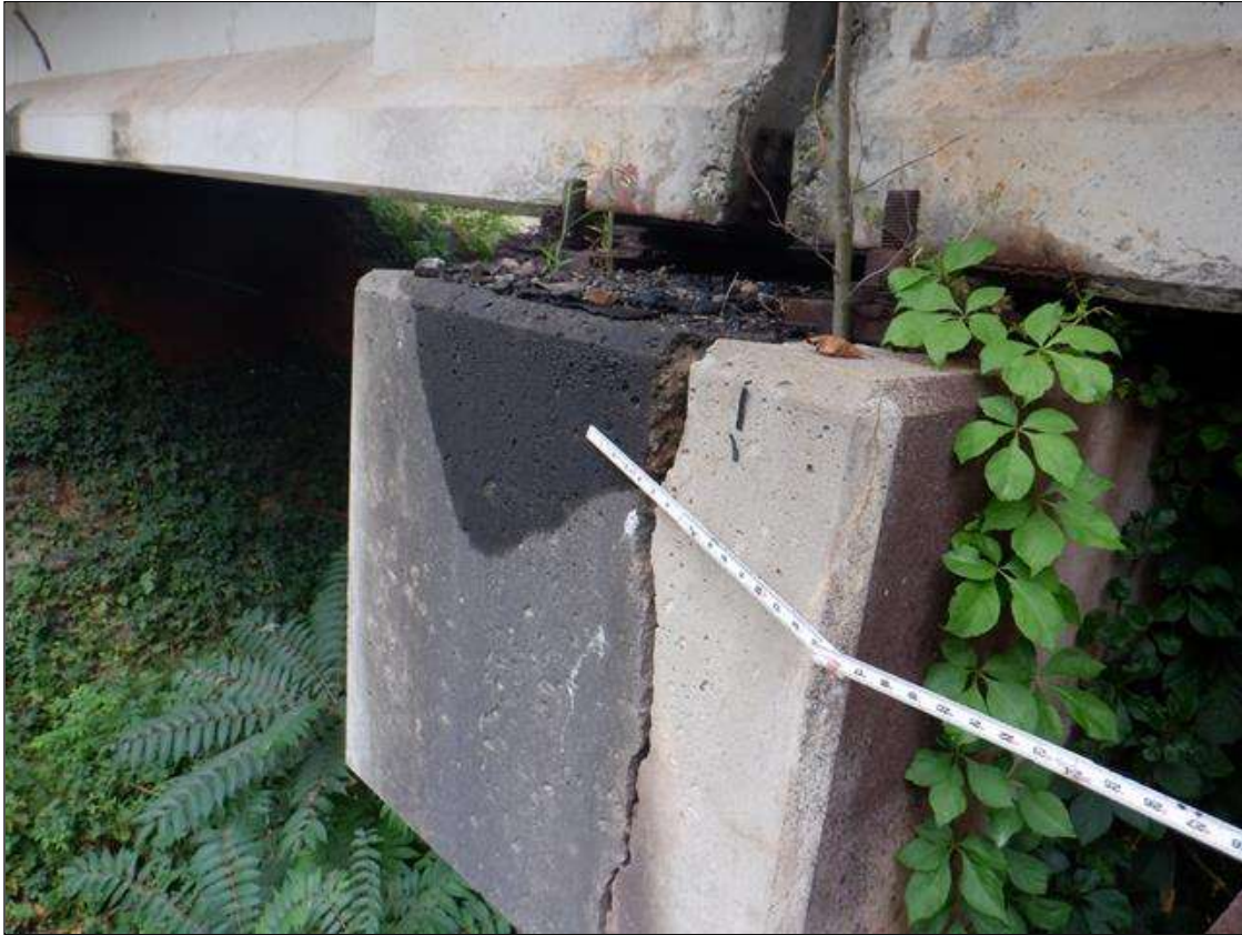
Bent 2 Cap 1: [PAR] along length, vertical crack [full height x up to 2-1/4in] traveling through all original bearing area; intermittently along length, delamination [up to full height]; along length multiple cracks [up to 20ft x up to 1/8in] with rust stain and efflorescence buildup; along top of South face, multiple spalls [6ft x 6in x 8in deep] with exposed primary and secondary rebar [up to 50% loss]; a replacement/crutch has been placed adjacent to original cap with the new bearing area 28in South of original; wood blocks have been placed in all bays over original bent 2 as additional support at concrete diaphragms
