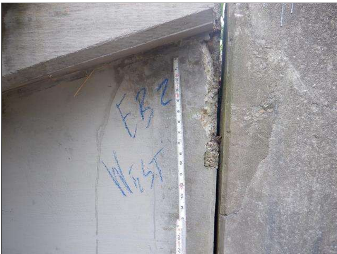
End bent 2 backwall: at West end, spall [12in x 4in x 1-1/2in deep]
