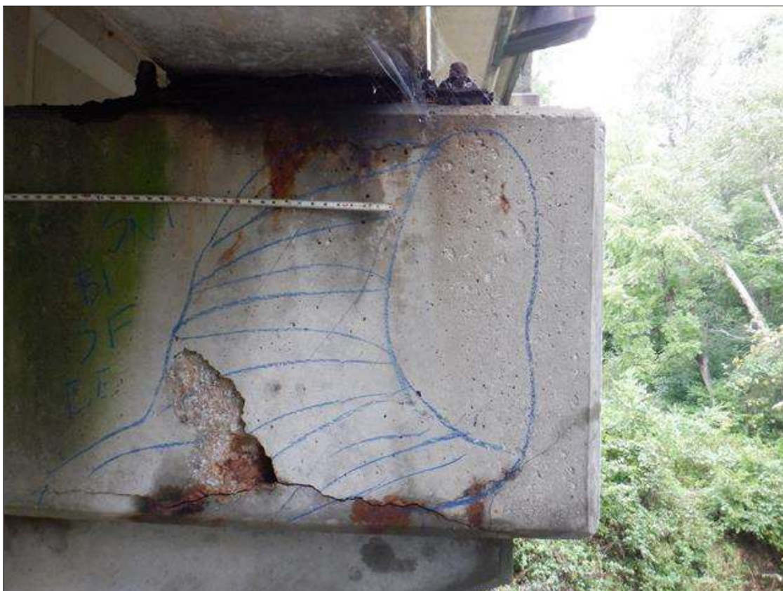
Bent 1 Cap 1: South face below girder 5, spall [40in x 30in x 1-1/4in deep] with exposed rusted reinforcing [loss up to 1/16in]
