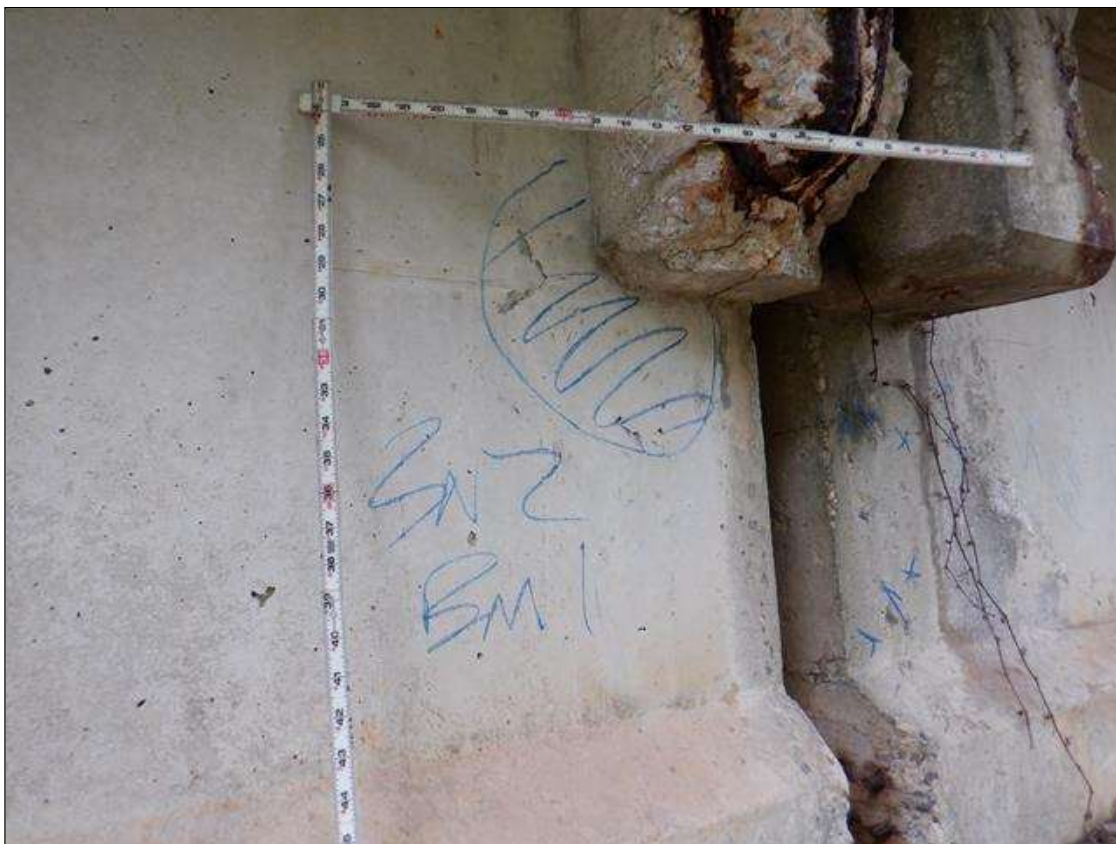
Span 2 Beam 1: West face at near end, delamination [11in x 10in]
