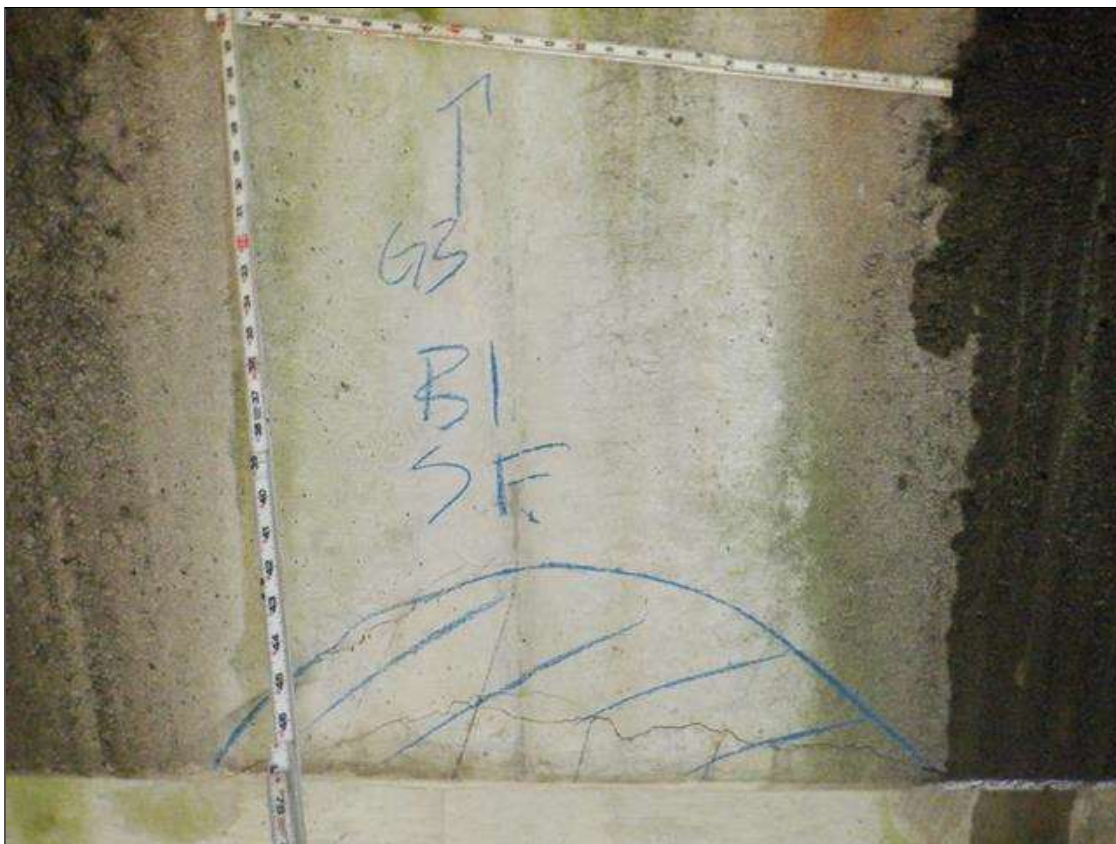
Bent 1 Cap 1: South face below girder 3 at bottom edge, delamination [30in x 10in]
