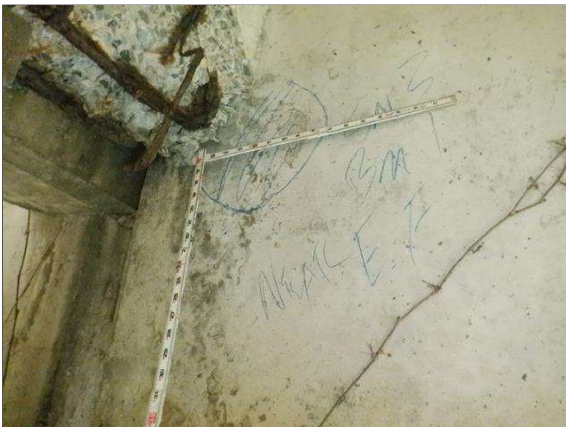
Span 3 Beam 1: East face at near end, delamination [10in diameter]
