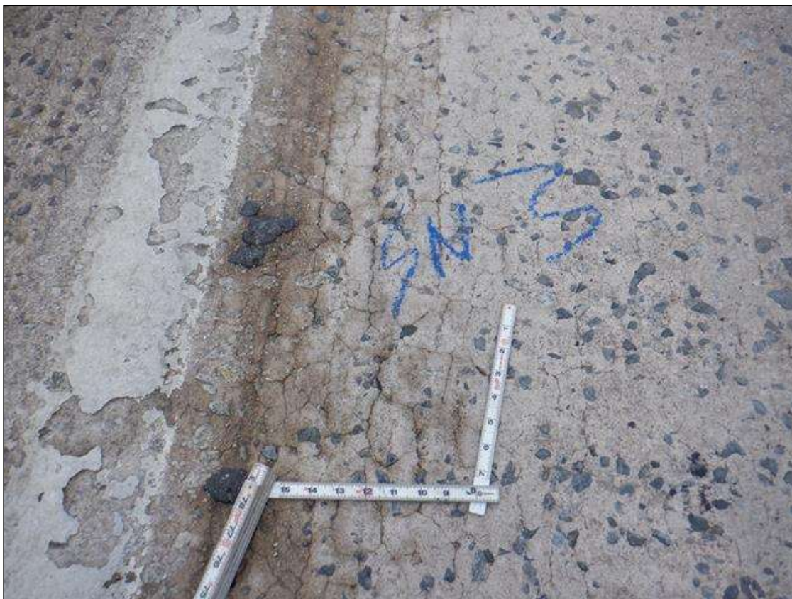
Span 3 Deck: throughout span, map cracking [up to 0.03in]
