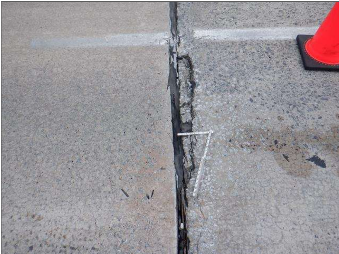
Span 3 Deck: [PAR] adjacent to joint over bent 2, spall/delamination [3ft x 5in x 2-1/2in deep]
