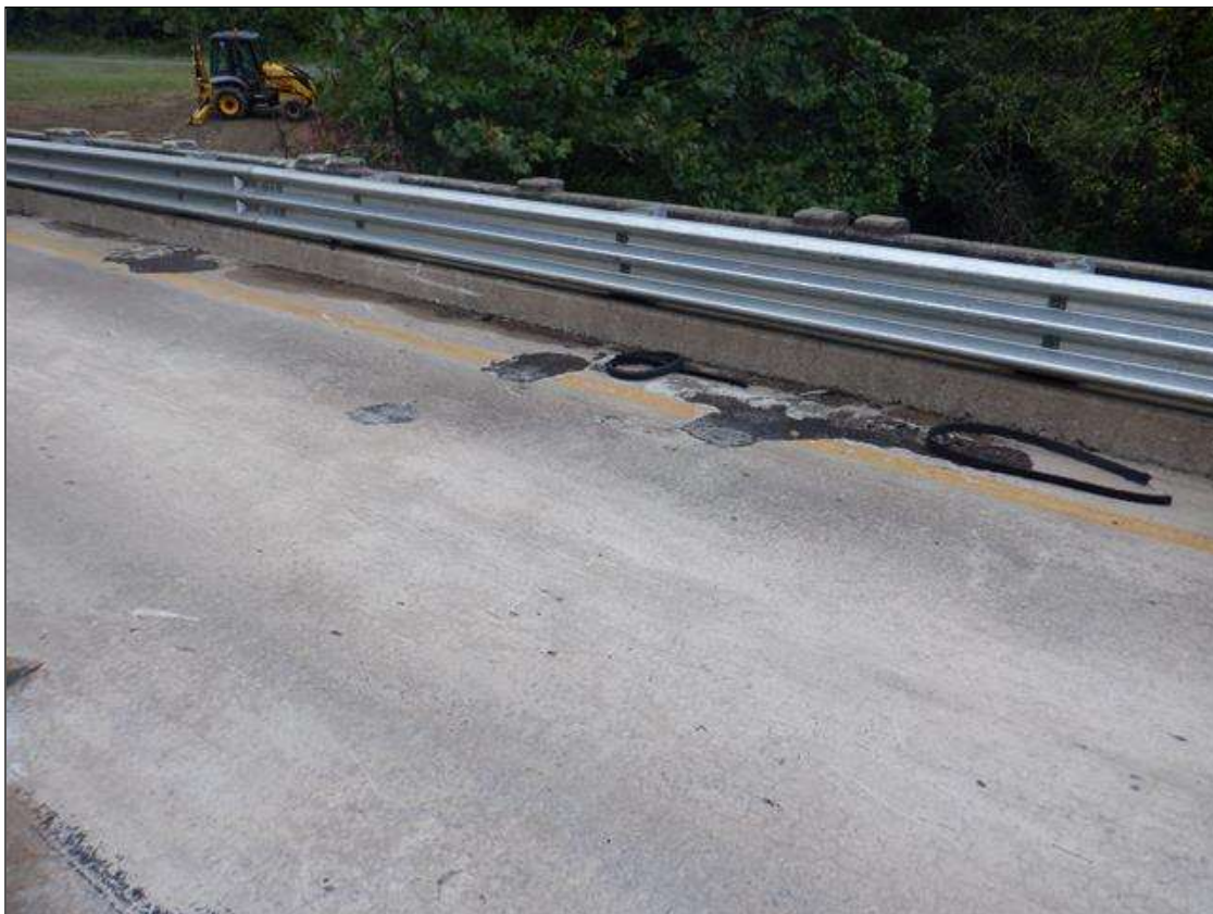
Span 2 Deck: at West shoulder 30ft from bent 2, sound patch [1ft-4in x 1ft-4in]
