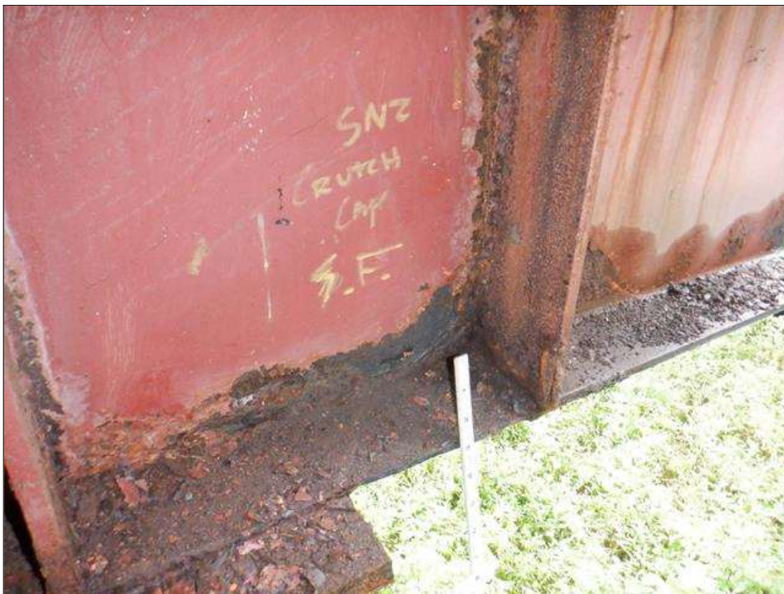
Bent 1 Cap 1: [PAR] below beam 5, active corrosion with section loss, bottom flange [16in x full width - 5/16in avg rem]; top flange [20in x full width - 7/16in avg rem]; lower web [16in x up to 2in - 1/4in avg rem]; web adjacent to East stiffener [full height x 1in - 1/4in avg rem]
