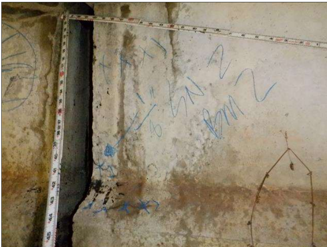
Span 2 Beam 2: [PAR] East face at near end, horizontal crack [3in x 1/8in]
