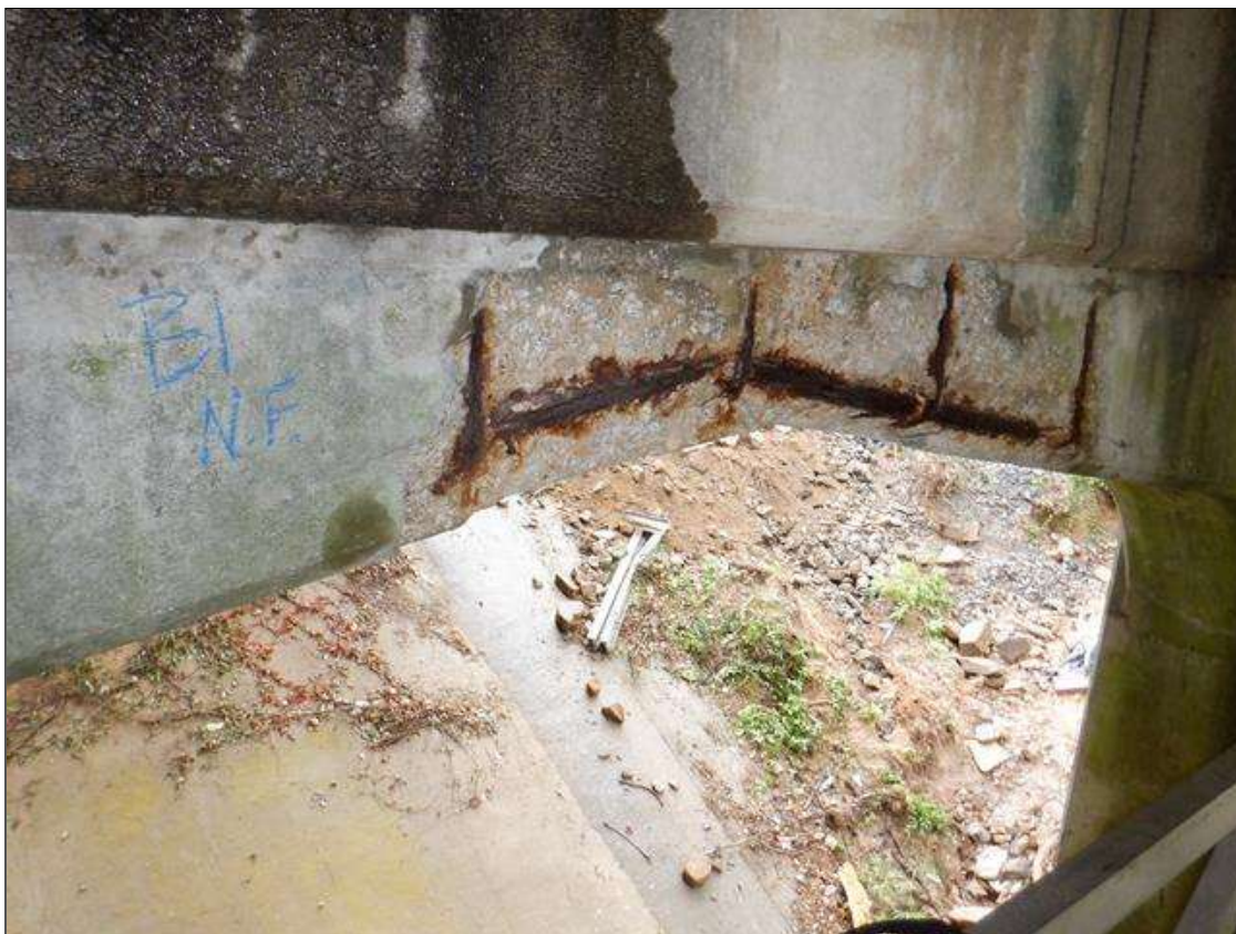
Bent 1: North face of center corbel below girder 3, spall/delamination [75in x 12in x 6in deep] with exposed rusted reinforcing [up to 100% loss]
