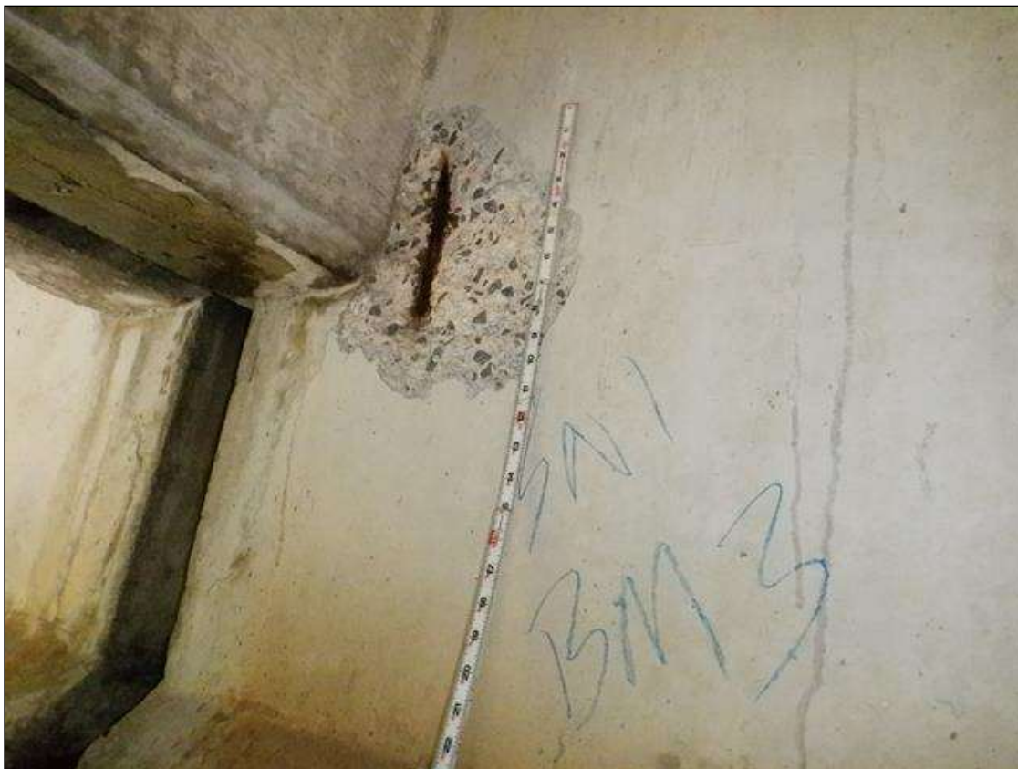
Span 1 Beam 3: [PAR] West face at far end, spall [13in x 10in x 1in deep] with exposed rusted reinforcing [up to 1/8in]
