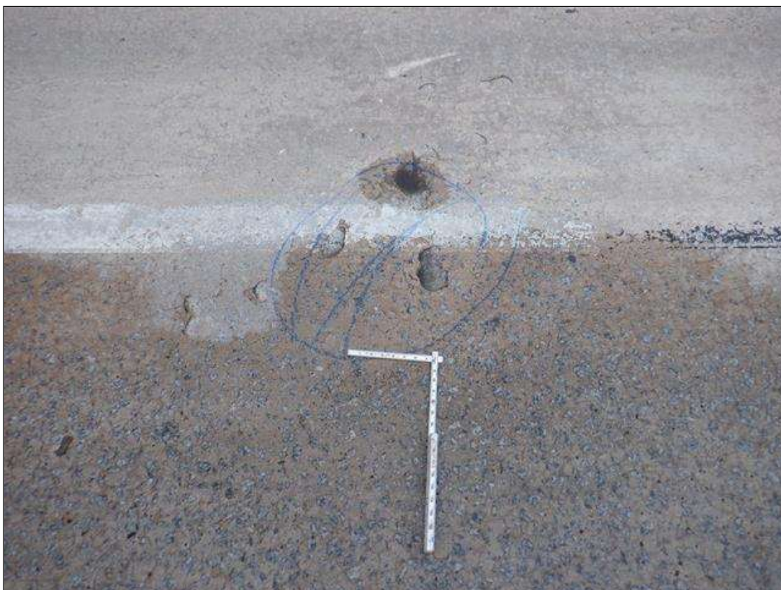
Span 2 Deck: at left lane near midspan, two [2] spall/delaminations [up to 2ft diameter x 1in deep]
