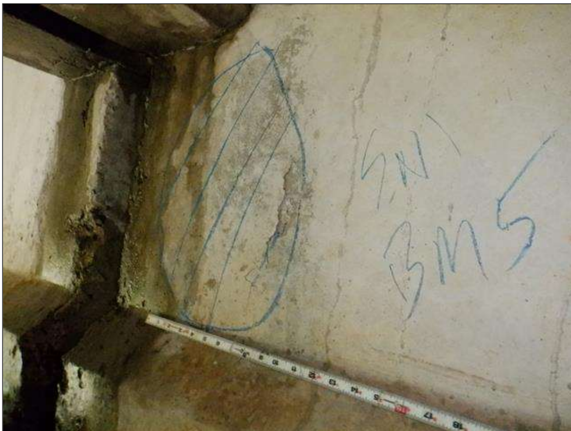
Span 1 Beam 5: West face at far end, delamination [11in x 15in]
