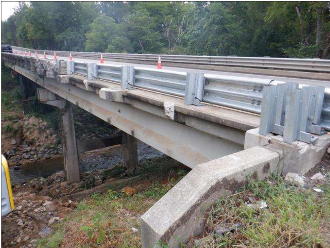
Span 1 Left Bridge Rail: [PAR] at near end, vehicular impact damage [2/3 of length missing], repair crew onsite at time of inspection
