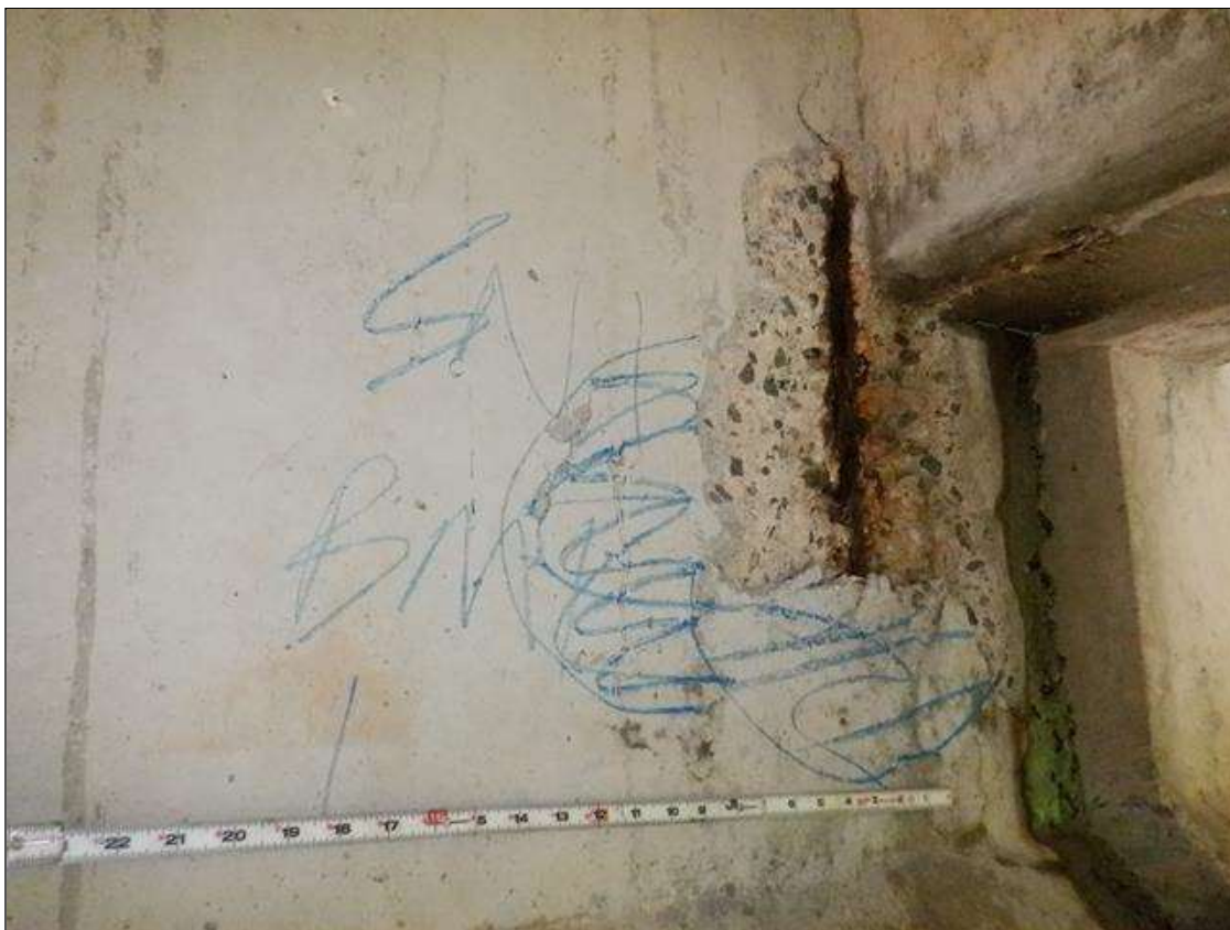
Span 1 Beam 1: [PAR] East face at far end, spall [18in x 21in x 1in deep] with exposed rusted reinforcing [up to 1/8in]
