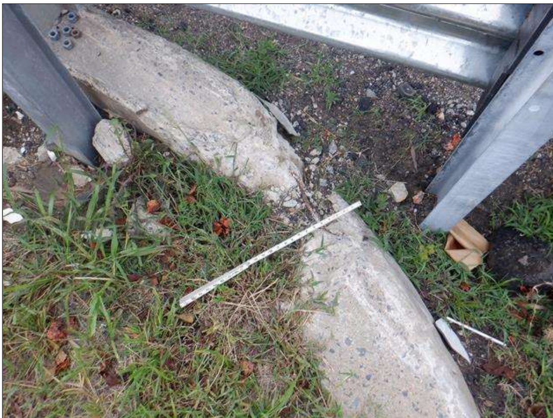
Southwest approach curb: vehicular impact damage [full length x full width x full depth] with exposed rusted reinforcing [loss < 1/16in]
