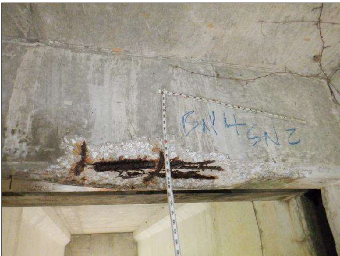
end diaphragm in bay 4 at bent 2, spall [5ft x 1ft x 4in deep] with exposed rusted reinforcing [loss up to 1/8in]
