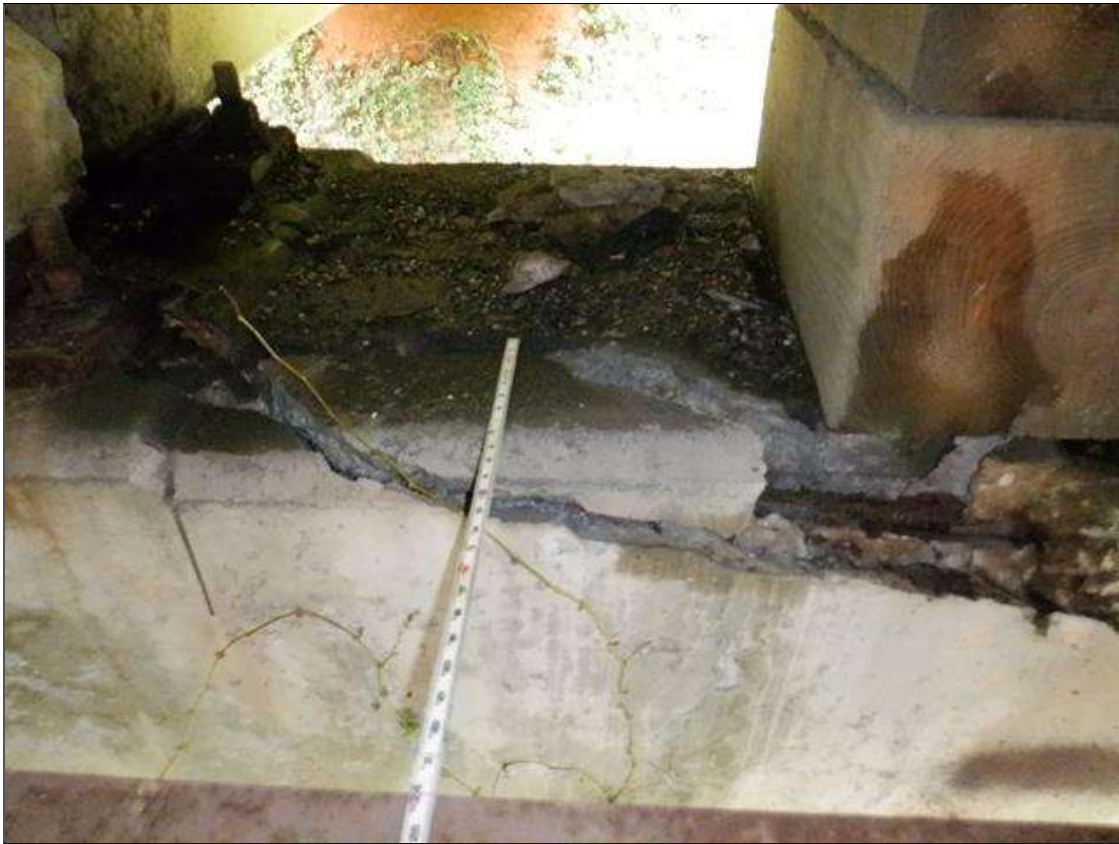
Bent 2 Cap 1: [PAR] along length, vertical crack [full height x up to 2-1/4in] traveling through all original bearing area; intermittently along length, delamination [up to full height]; along length multiple cracks [up to 20ft x up to 1/8in] with rust stain and efflorescence buildup; along top of South face, multiple spalls [6ft x 6in x 8in deep] with exposed primary and secondary rebar [up to 50% loss]; a replacement/crutch has been placed adjacent to original cap with the new bearing area 28in South of original; wood blocks have been placed in all bays over original bent 2 as additional support at concrete diaphragms
