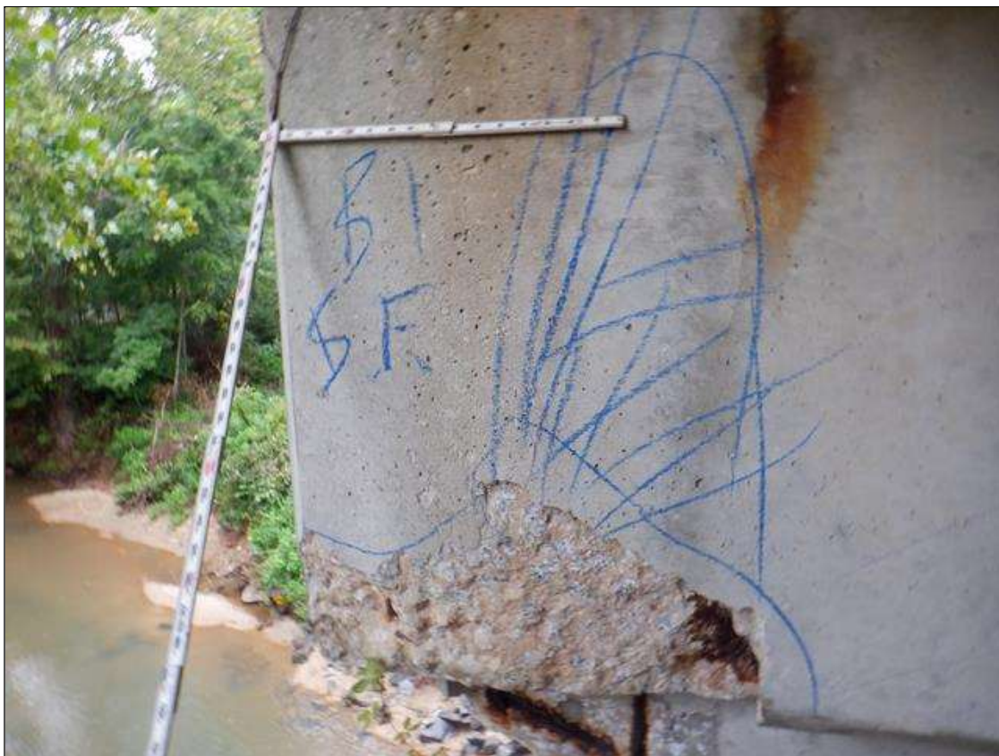
Bent 1 Cap 1: South face below West overhang, spall [40in x 27in x 3in deep] with exposed rusted reinforcing [loss up to 1/8in]
