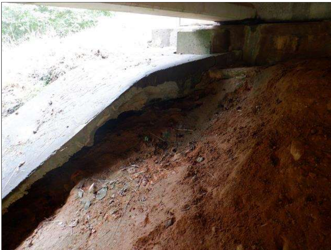
Slope Protection: below concrete gutter below span 1 East overhang, erosion [full length x 2ft x 3ft deep]
