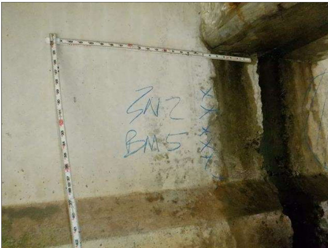
Span 2 Beam 5: West face at near end, vertical crack [14in x hairline]
