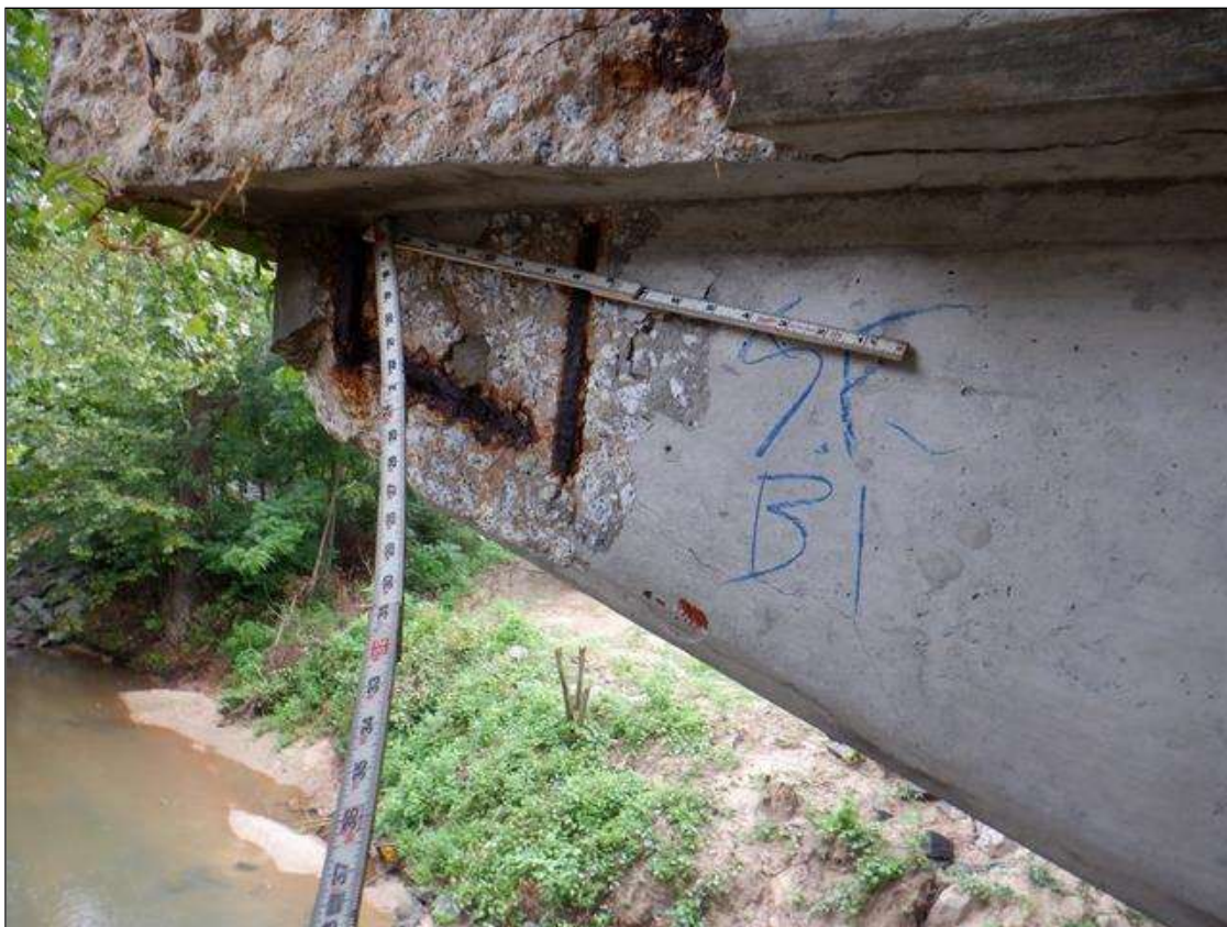
Bent 1: South face of West corbel adjacent to column 1, spall [16in x 10in x 2in deep] with exposed rusted reinforcing [loss up to 1/8in]
