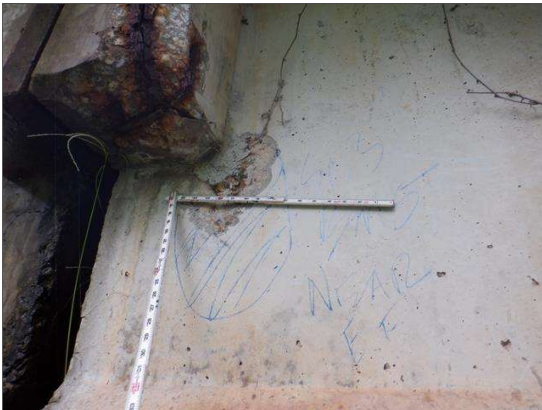
Span 3 Beam 5: East face at near end, spall/delamination [15in x 9in x 1/2in deep]
