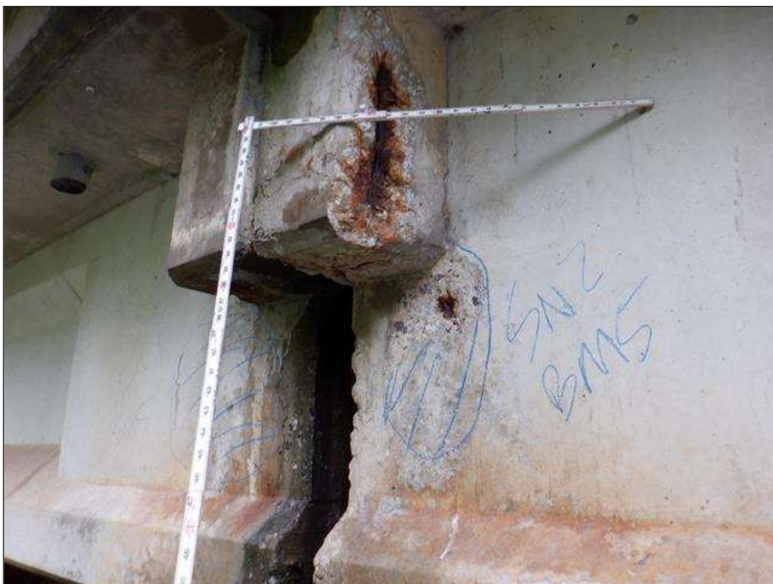
Span 2 Beam 5: East face at near end, spall/delamination [8in x 12in x up to 1in deep] with exposed rusted reinforcing [loss up to 1/16in]
