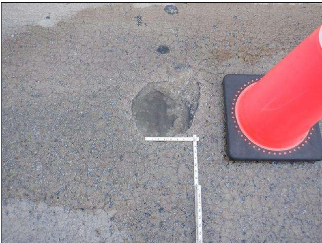
Span 1 Deck: centerline of roadway near midspan, spall [10in diameter x 1in deep] with exposed rusted reinforcing [no loss]
