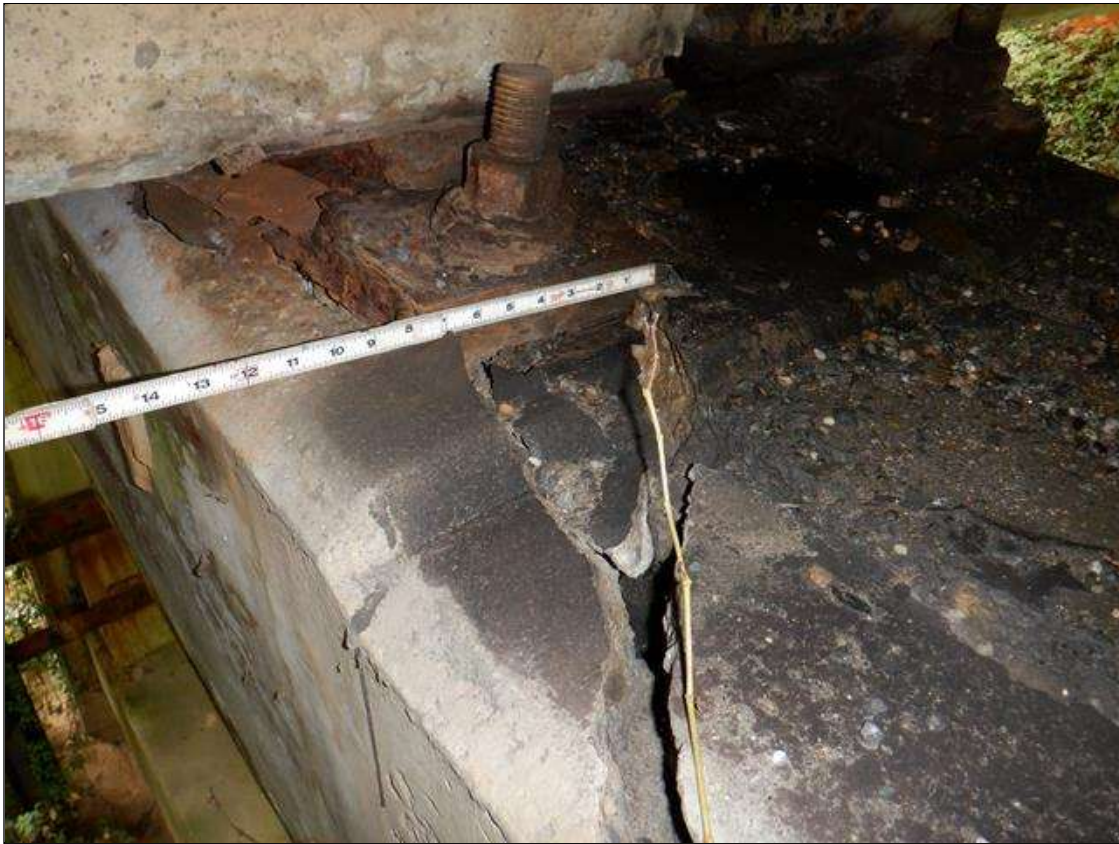
Bent 2 Cap 1: [PAR] along length, vertical crack [full height x up to 2-1/4in] traveling through all original bearing area; intermittently along length, delamination [up to full height]; along length multiple cracks [up to 20ft x up to 1/8in] with rust stain and efflorescence buildup; along top of South face, multiple spalls [6ft x 6in x 8in deep] with exposed primary and secondary rebar [up to 50% loss]; a replacement/crutch has been placed adjacent to original cap with the new bearing area 28in South of original; wood blocks have been placed in all bays over original bent 2 as additional support at concrete diaphragms
