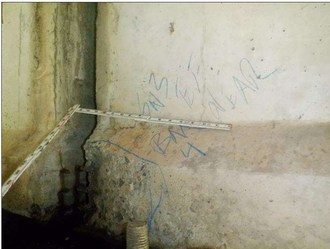
Span 3 Beam 4: [PAR] East face bottom flange at near end, spall [8in x 10in x 2in deep], with three [3] exposed prestress strands [loss up to 1/16in]
