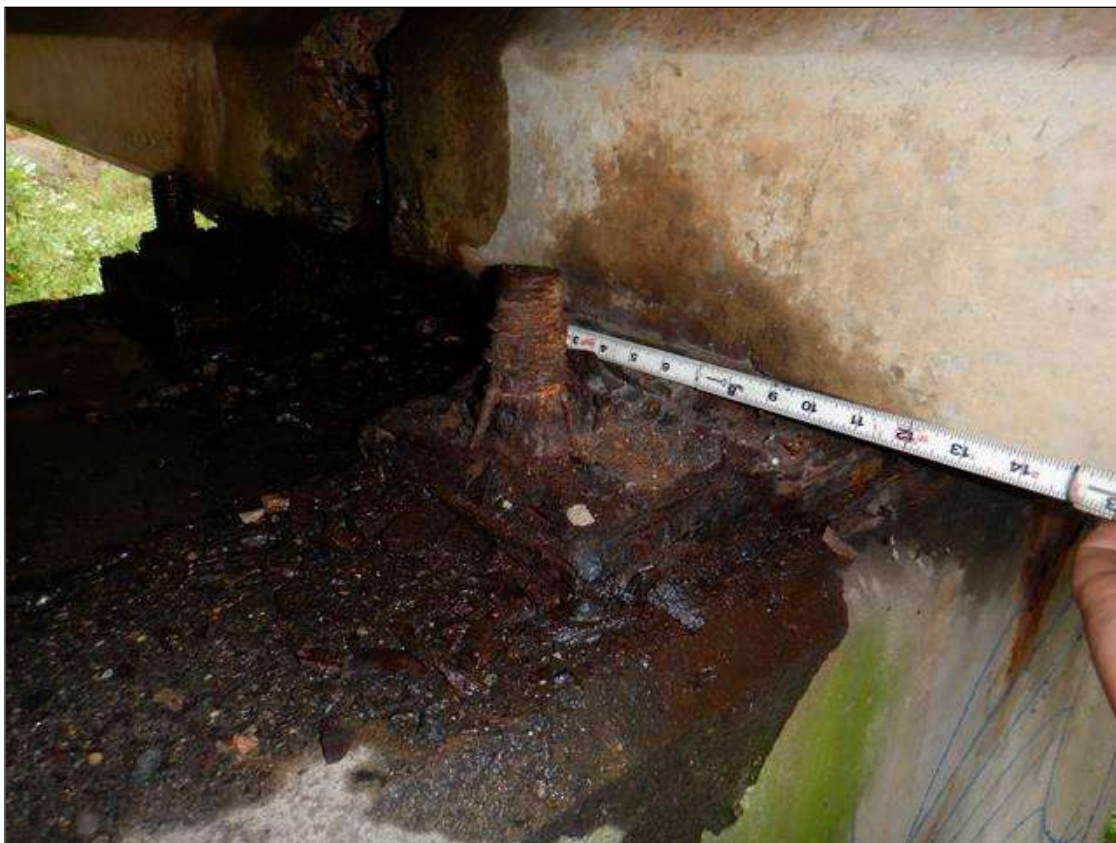
Span 1 Beam 5 Far Bearing: active corrosion with section loss [up to 1/4in] with section loss on anchor bolts & nuts [up to 50%]
