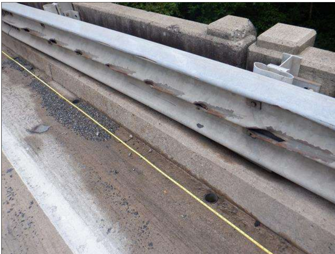
Span 3 Right Bridge Rail: along length, vehicular impact damage [23ft] with scrapes and gauges
