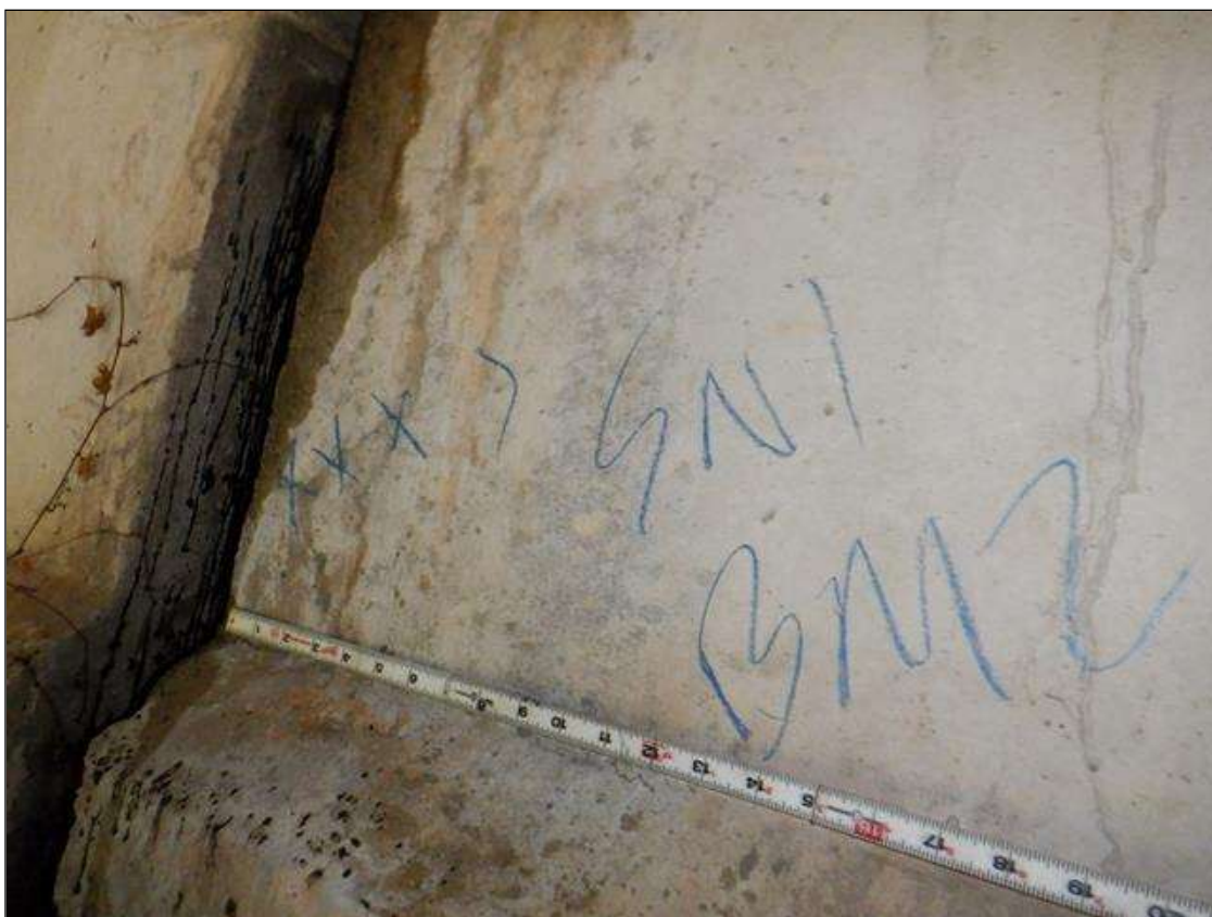
Span 1 Beam 2: West face at far end, diagonal crack [8in x 0.009in]
