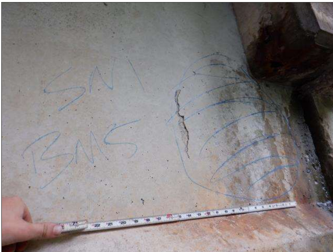
Span 1 Beam 5: East face at far end, delamination [17in diameter]
