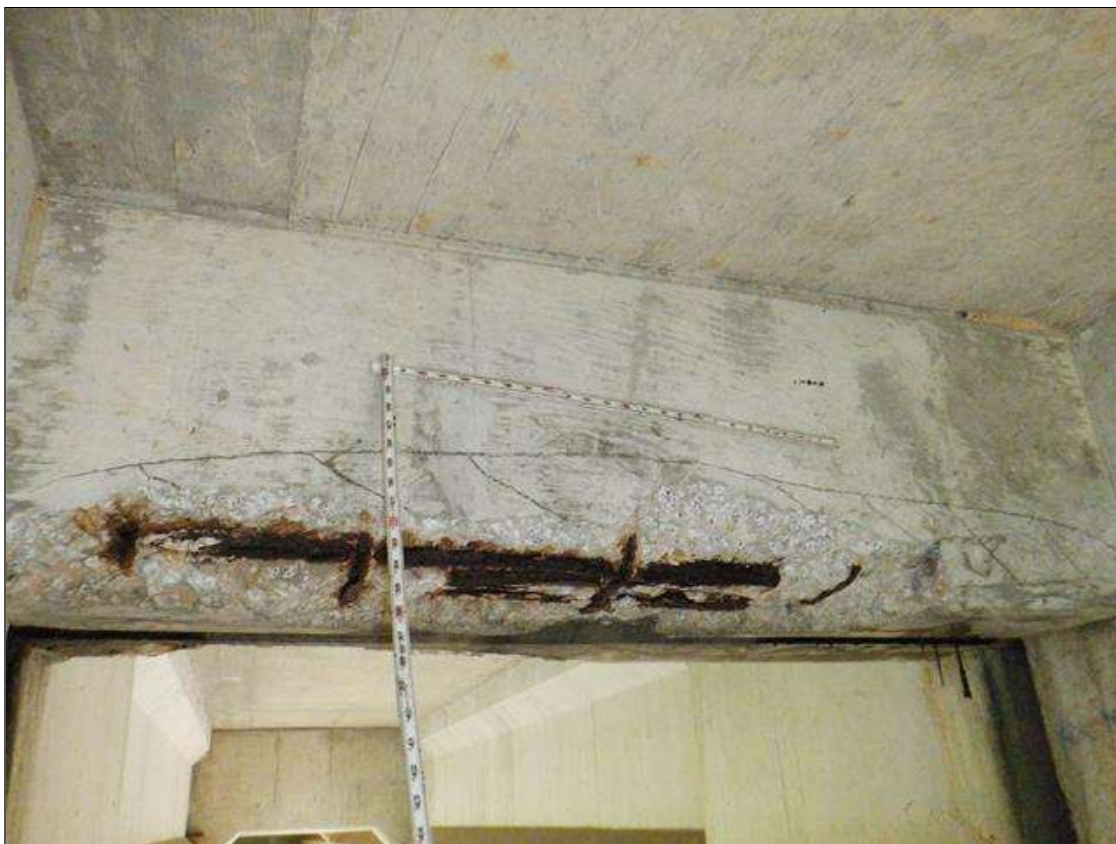
end diaphragm in bay 3 at bent 2, spall [5ft x 1ft x 4in deep] with exposed rusted reinforcing [loss up to 1/8in]
