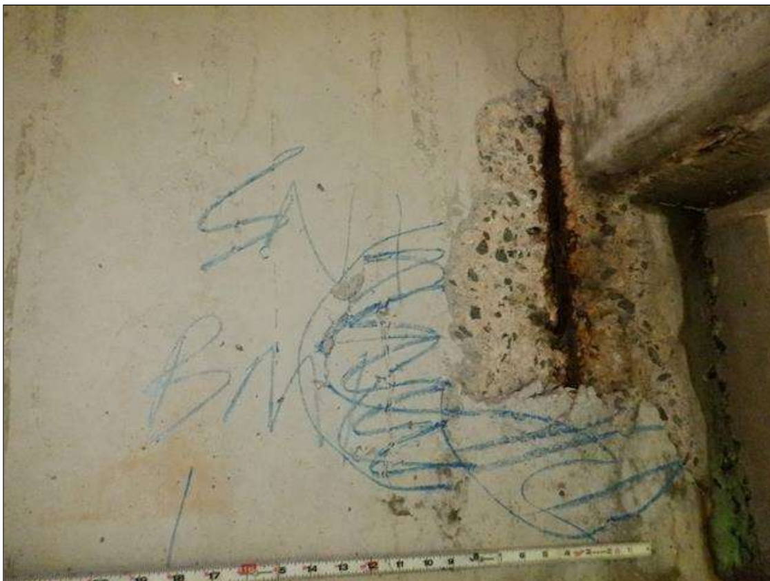
Span 1 Beam 1: [PAR] East face at far end, spall [18in x 21in x 1in deep] with exposed rusted reinforcing [up to 1/8in]
