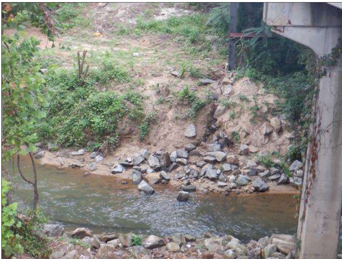
at upstream, dwnstream, and channel under bridge, cut banks [up to 8ft vertical]
