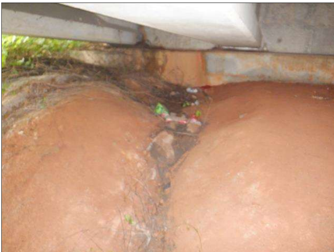
Slope Protection: at end bent 2, area of erosion [8ft x 20ft x up to 2ft deep]
