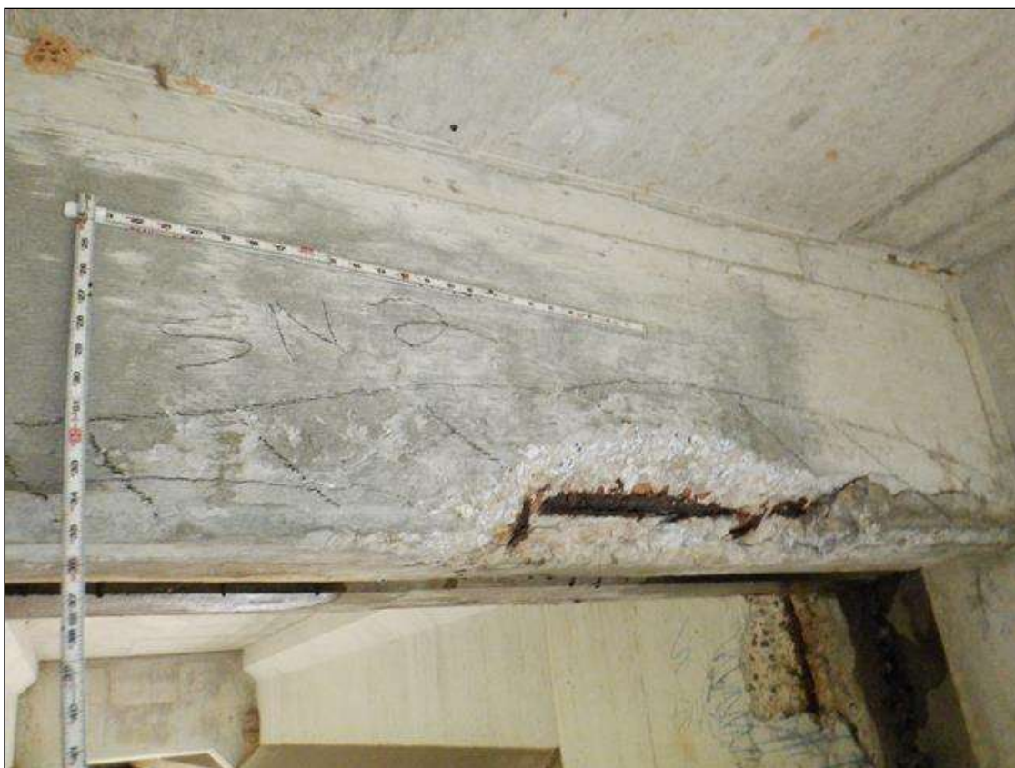
end diaphragm in bay 2 at bent 2, spall [5ft x 1ft x 4in deep] with exposed rusted reinforcing [loss up to 1/8in]
