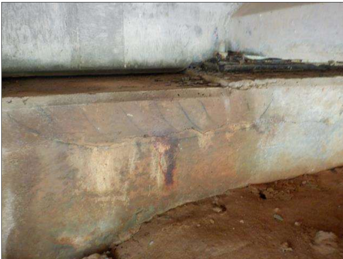
End Bent 1 Cap 1: below girder 4, delamination [3ft x 7in]
