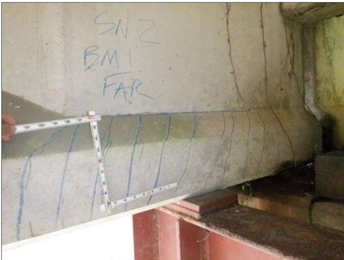
Span 2 Beam 1: bottom right flange at crutch bent, delamination [50in x 10in x 3in]
