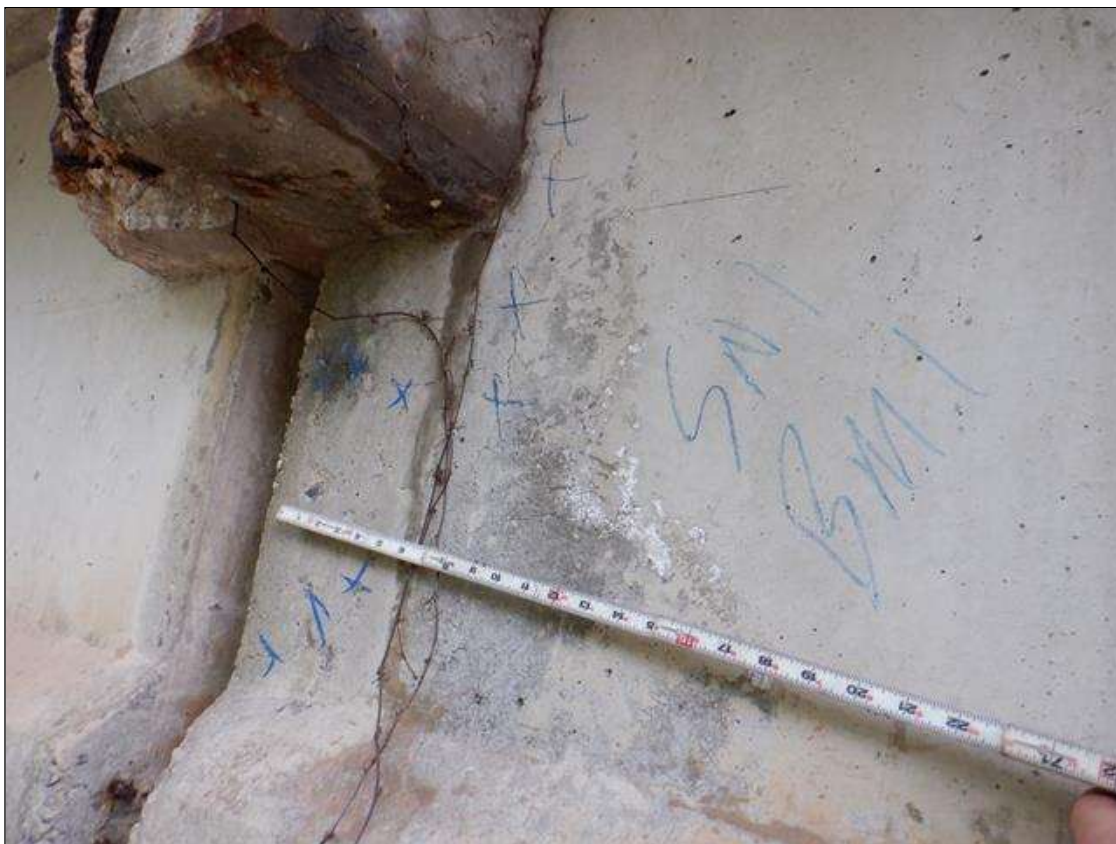
Span 1 Beam 1: West face at far end, multiple horizontal, vertical, and diagonal cracks [up to 18in x up to 0.004in]
