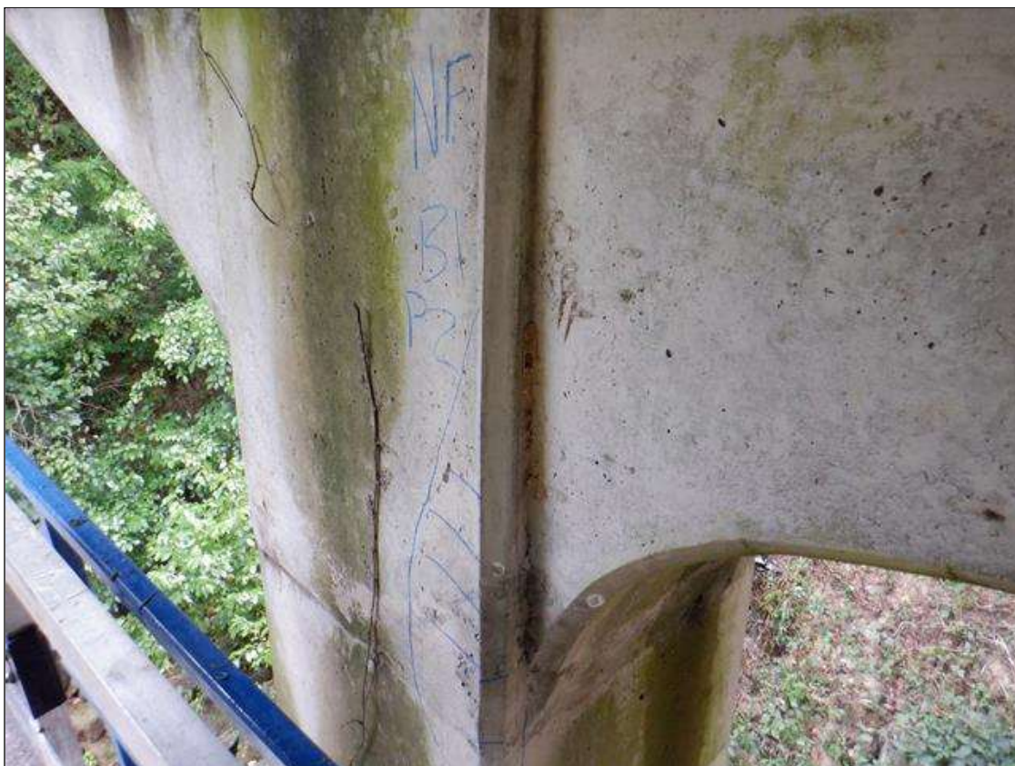
Bent 1 Pile 2: Northwest corner adjacent to corbel, delamination [20in x 7in]
