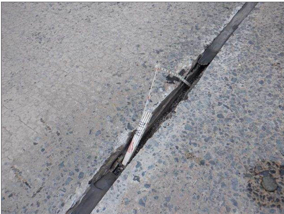
Expansion Joint : along length, areas of seal adhesion failure [full depth]
