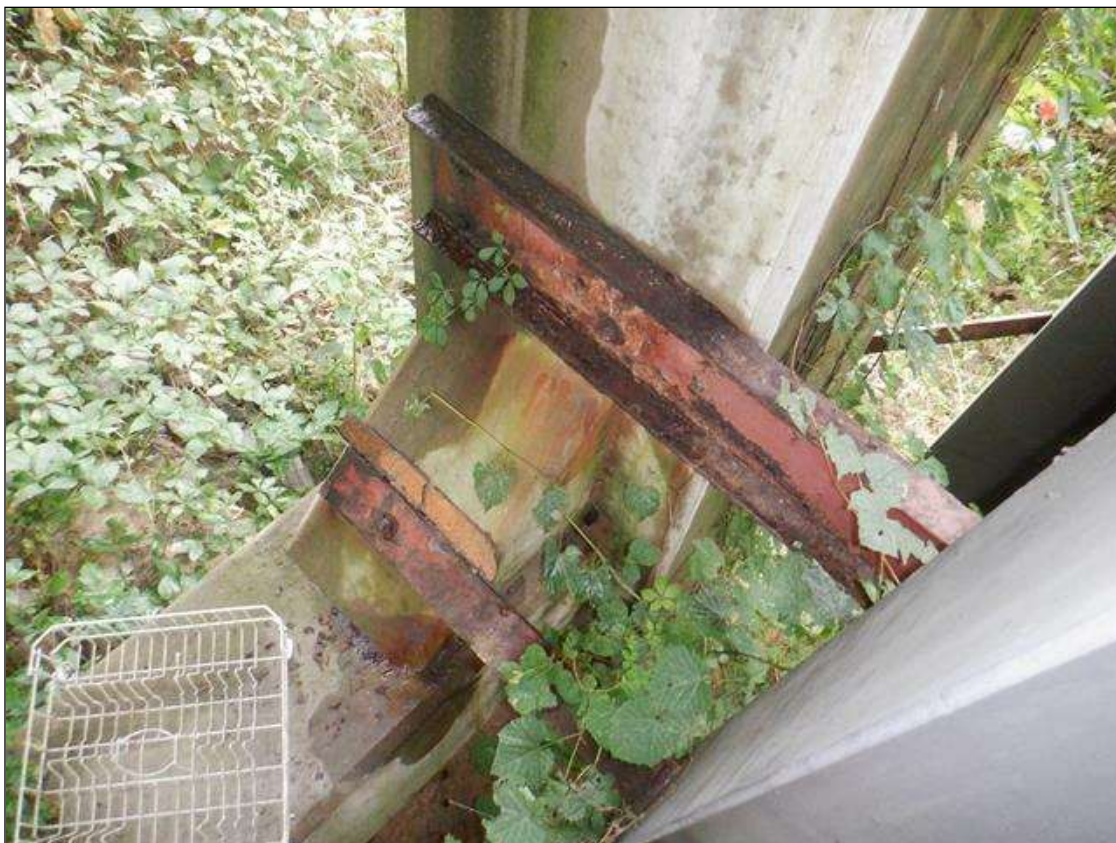
Crutch Bent: at metal angles and bracing attaching crutch bent to original bent 2, active corrosion with section loss [up to 1/8in]
