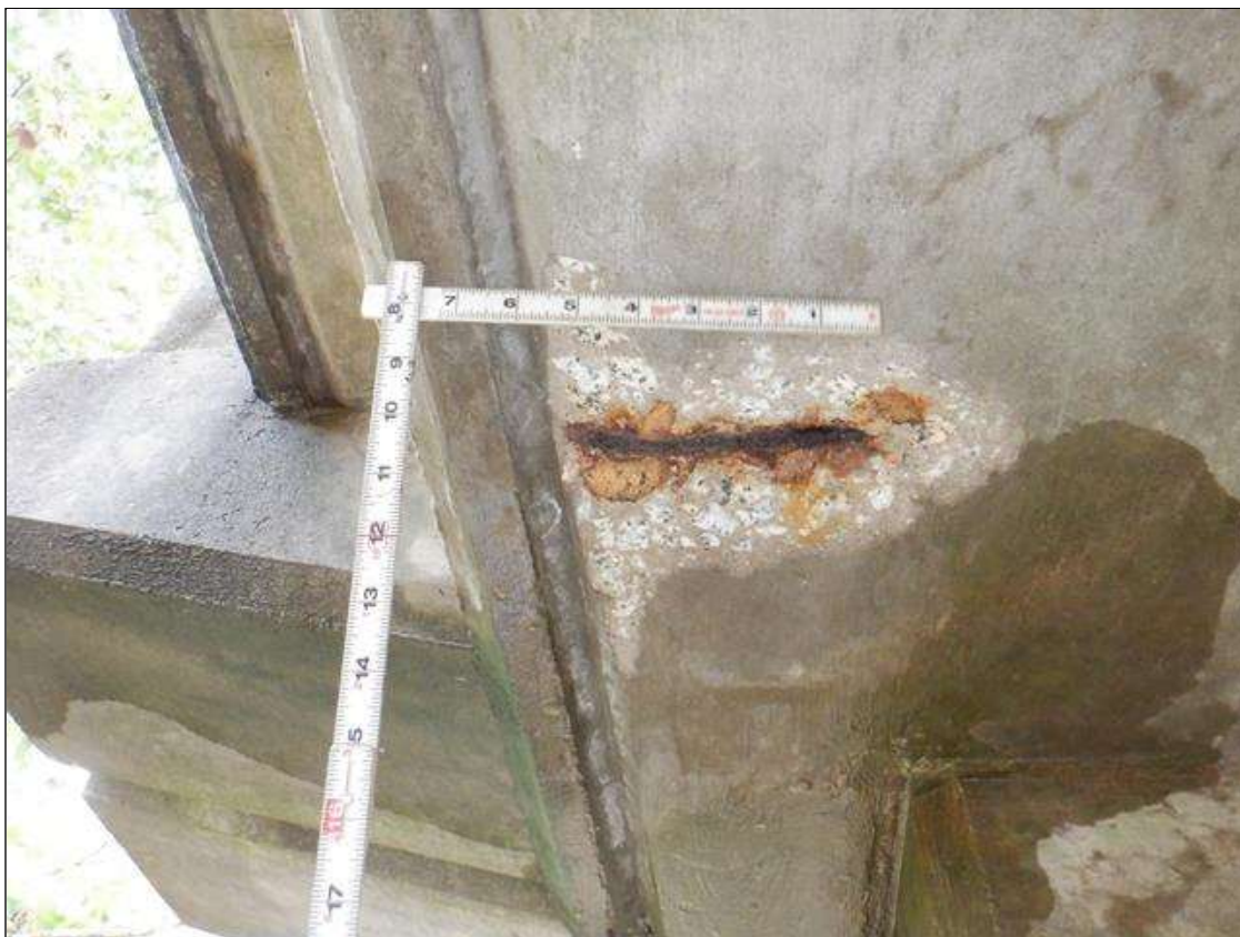
Span 1 Deck: underside West overhang at bent 1, spall [8in x 3in x 1/2in deep] with exposed rusted reinforcing [loss < 1/16in]
