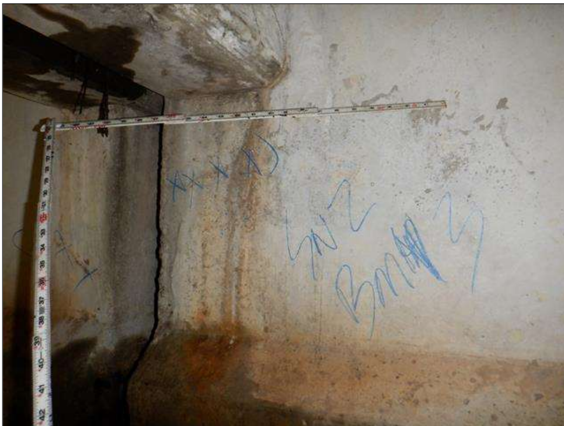
Span 2 Beam 3: West face at near end, three [3] horizontal cracks [up to 10in x hairline]
