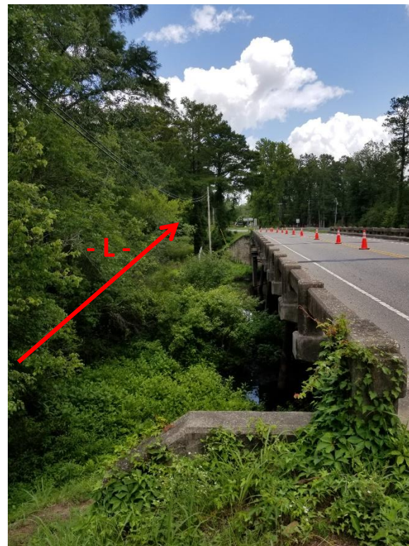
Photograph No. 2: View from existing End Bent 1 looking east at proposed End Bent 2
