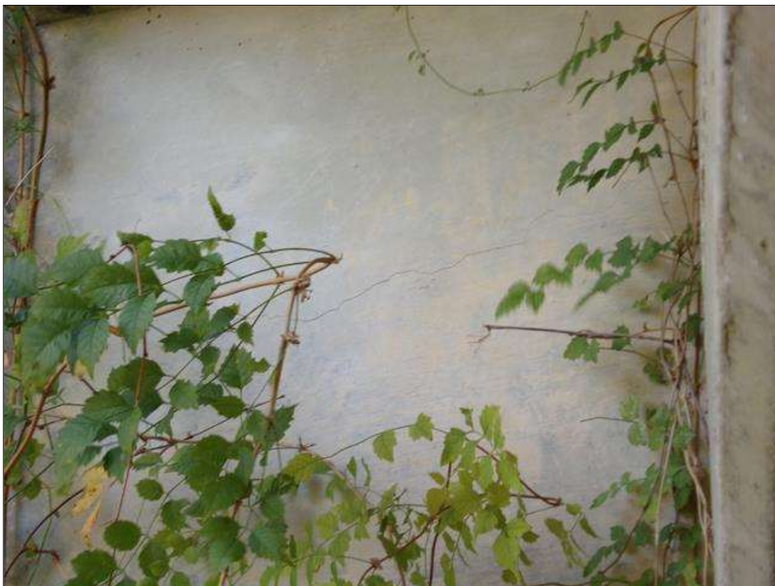
End Bent 2 Abutment: (2) UP TO 6 FEET X 1/64 INCHES HORIZONTAL CRACKS AT NORTH END
