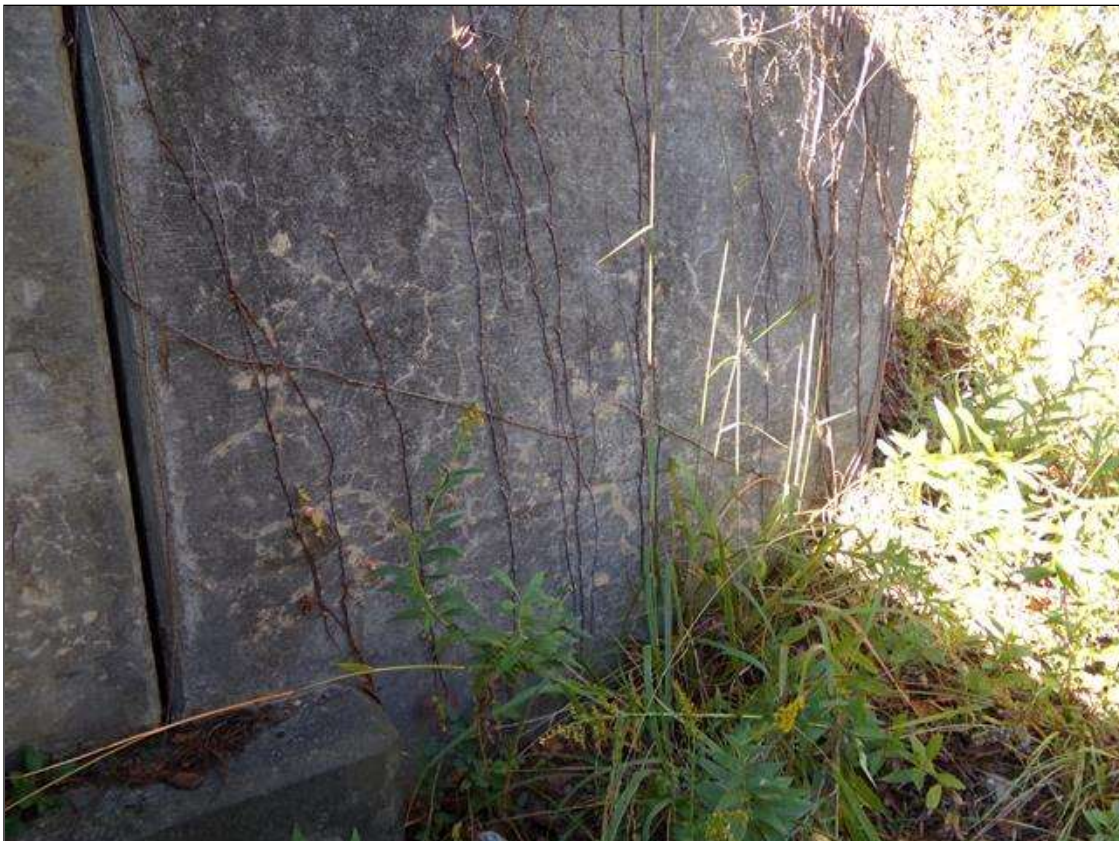
4 FEET X 4 FEET AREA OF HAIRLINE MAP CRACKING WITH EFFLORESCENCE ON NORTHWEST WINGWALL
