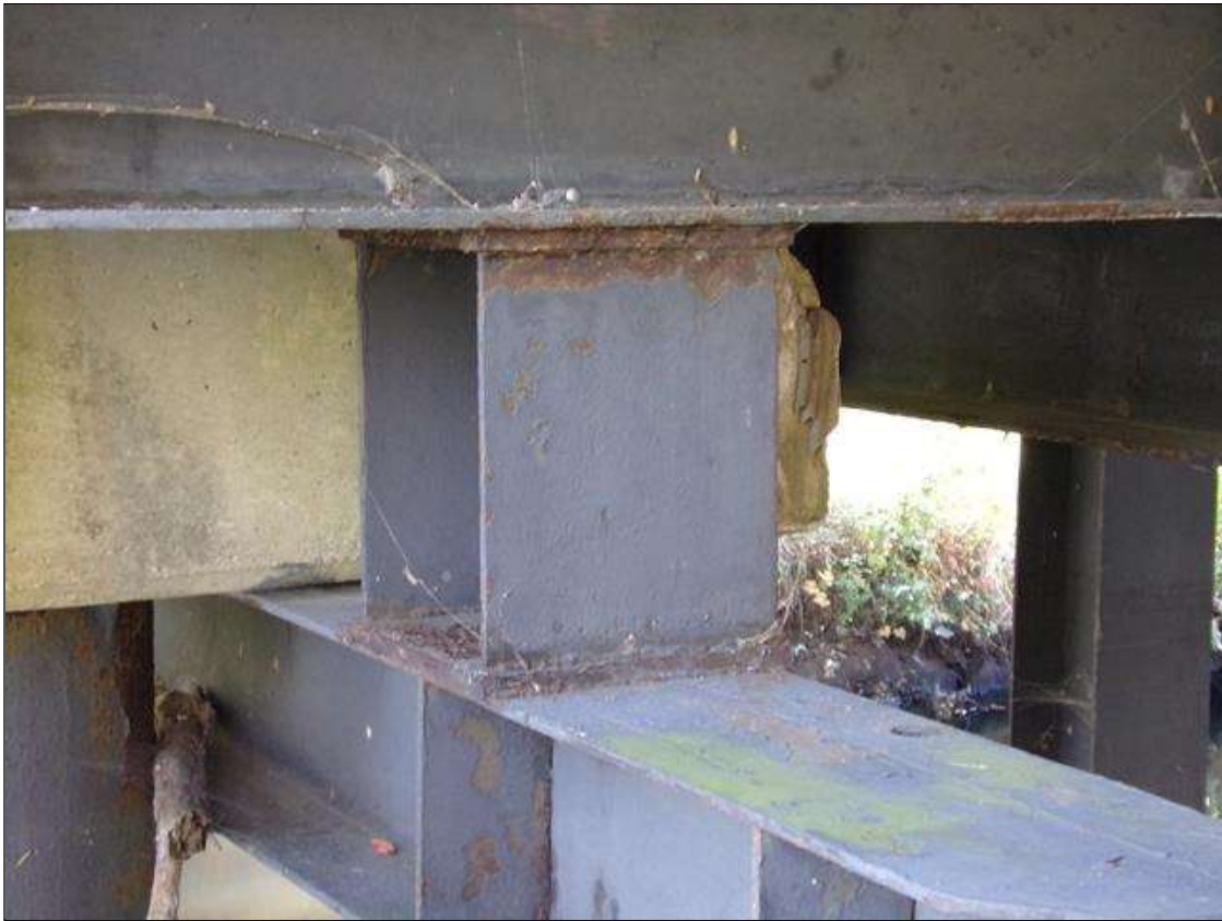
Bent 3 Row 1 Pile 1: 8 FEET OF FRECKLED RUST WITH ISOLATED LOCATIONS OF SURFACE RUST AT RANDOM THROUGHOUT.
