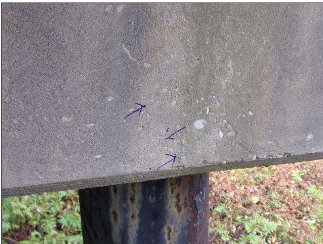
Bent 1 Cap 1: 6 INCHES X 1/64 INCHES DIAGONAL CRACK ON EAST FACE BENEATH BEAM 1.
