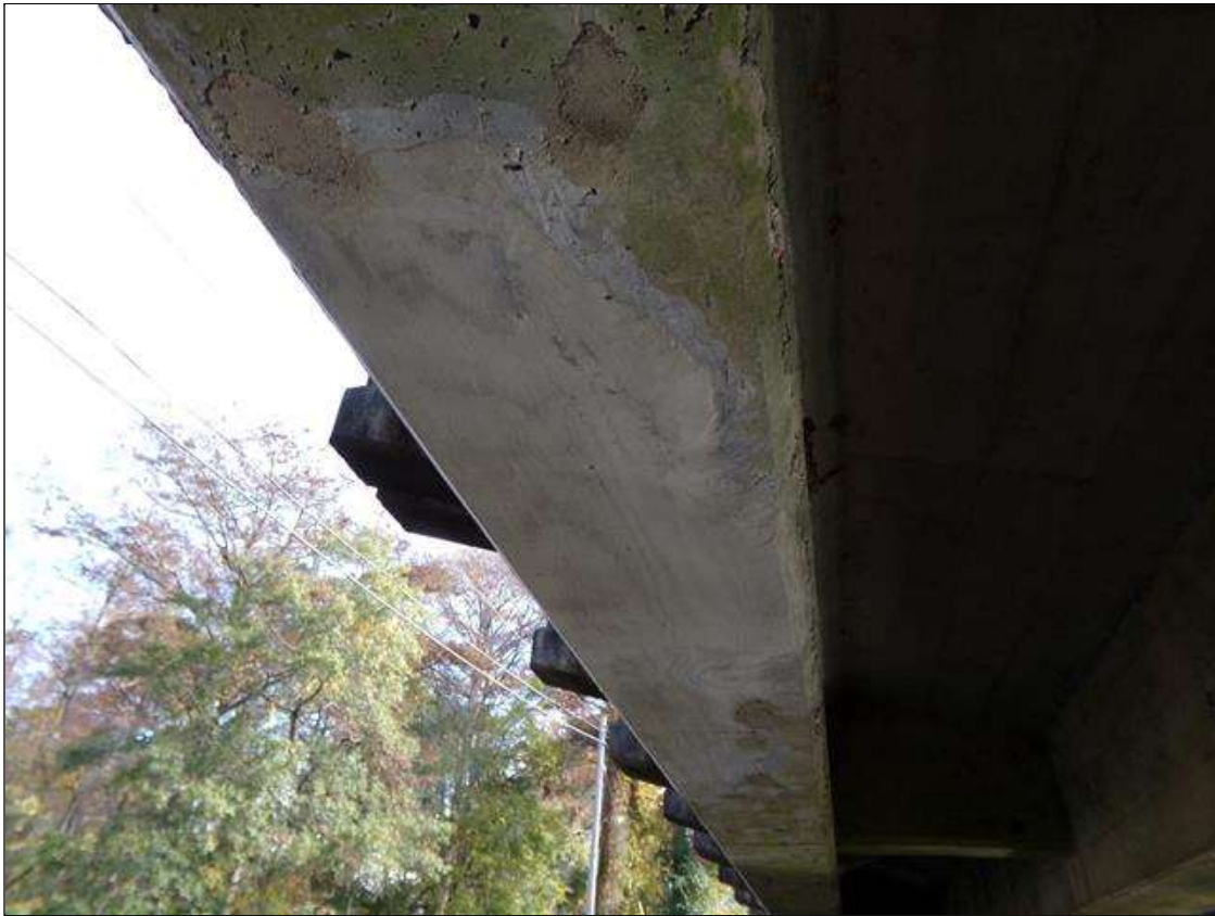
SPAN 3 Beam 1: 70 INCHES X 3 INCHES X UP TO 4 INCHES SPALL WITH EXPOSED REINFORCING ON THE SOUTH BOTTOM CORNER, 8 FEET FROM BENT 2.(PATCHED)
