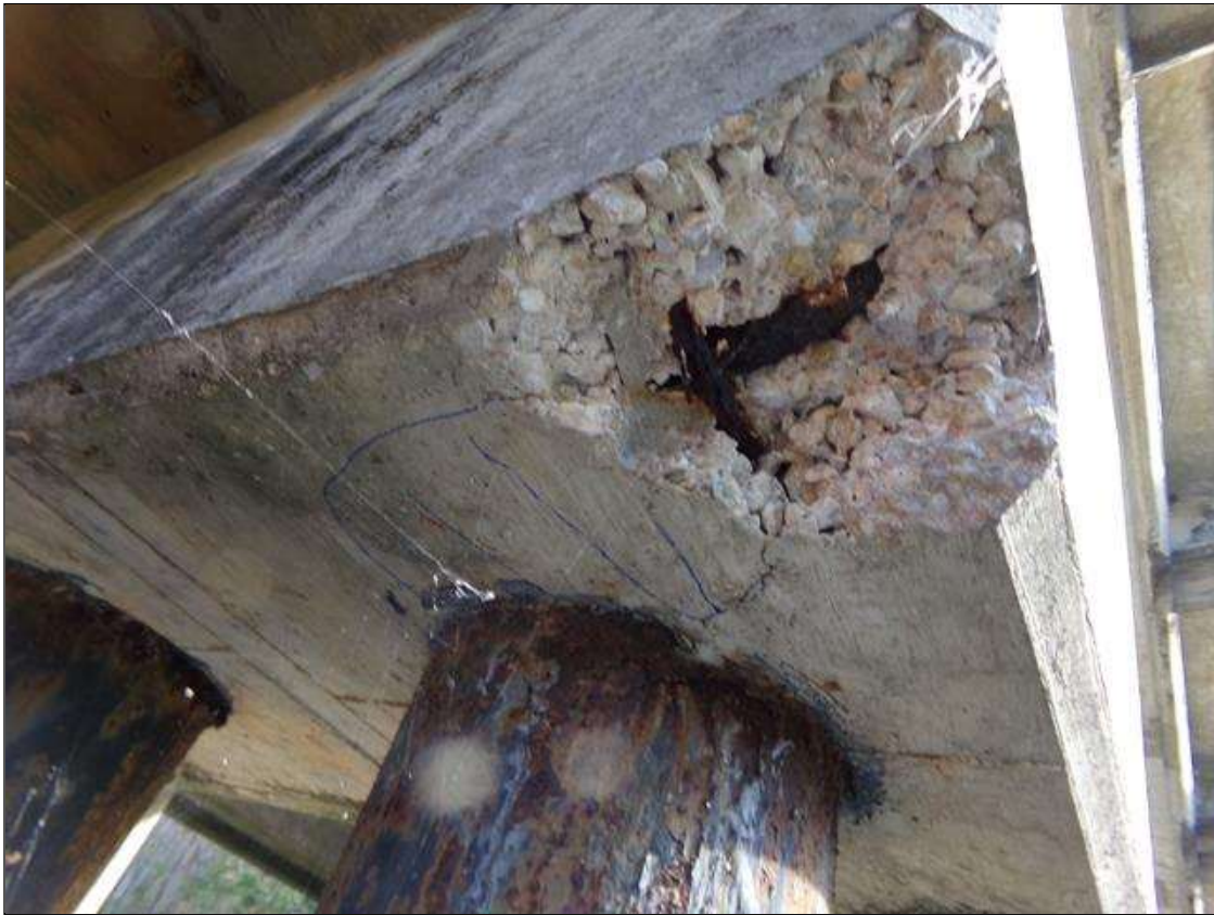
Bent 2 Cap 1: 19 INCH X 12 INCH X 4 INCH DEEP SPALL WITH EXPOSED REINFORCING AND AREA OF DELAMINATION ON SOUTHWEST BOTTOM CORNER (PAR)
