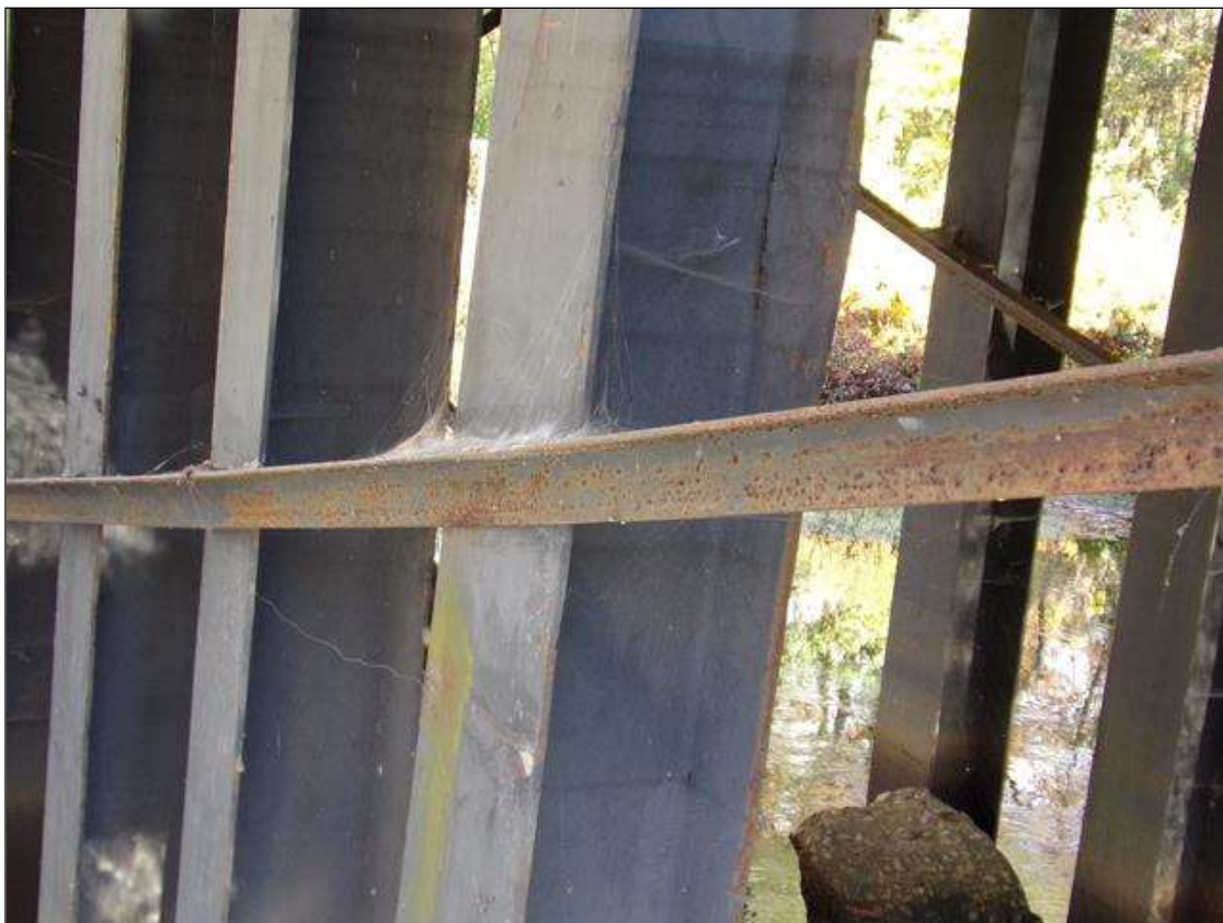
Bent 3 Row 1 Pile 1: 35 FEET OF SURFACE RUST ON WEST CROSS BRACING.
