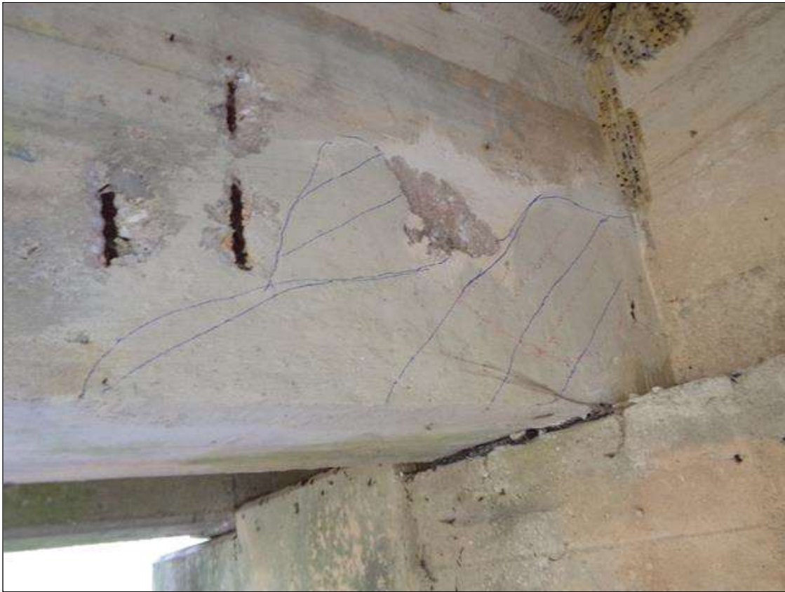
SPAN 2 Beam 2: 8 INCHES X 6 INCHES X 1 INCHES DEEP SPALL WITH ASSOCIATED 38 INCHES X 16 INCHES DELAMINATION ON SOUTH FACE AT BENT 2.
