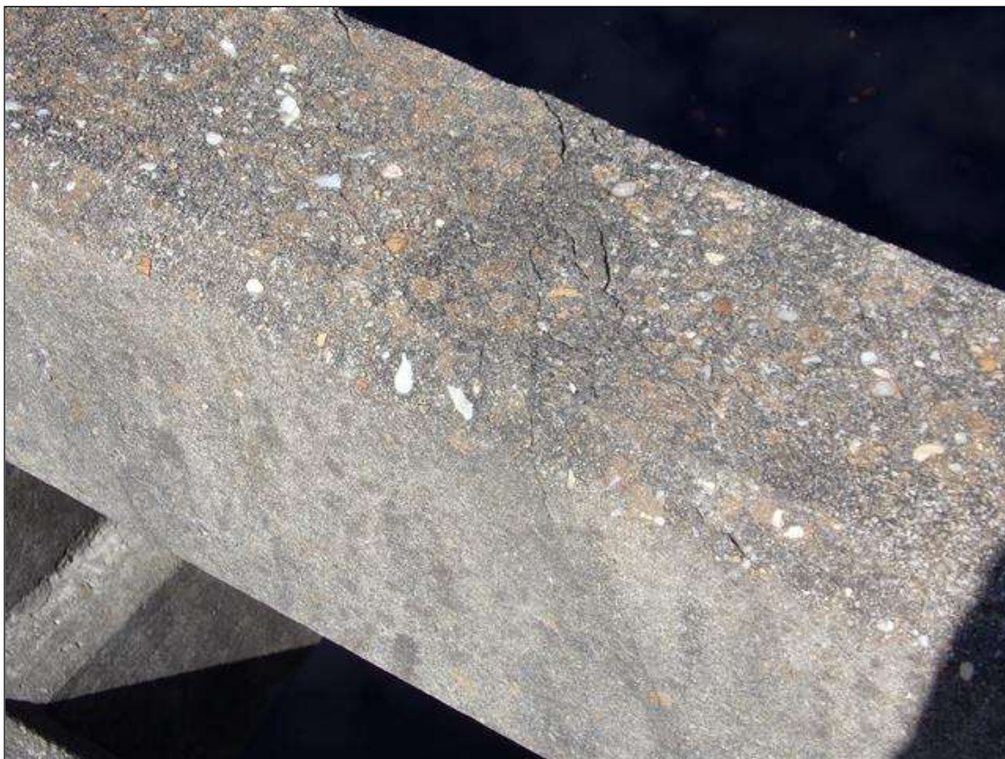
SPAN 4 Left Bridge Rail: (4) UP TO 1/16 INCHES CRACKS ON TOP AND NORTH FACE, 18 FEET FROM END BENT
