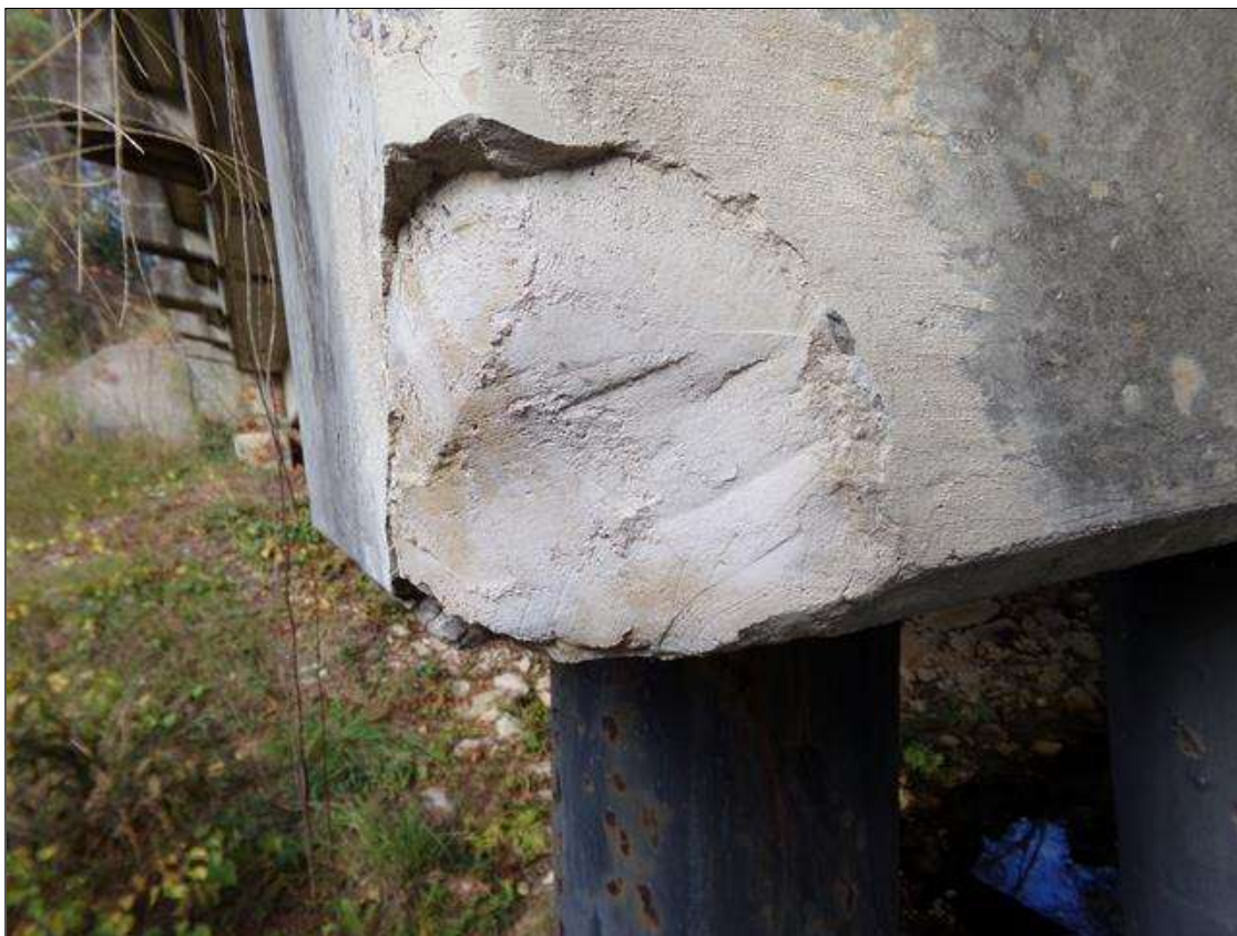
Bent 1 Cap 1: 8" X 7" X 5" DEEP SPALL IN THE SOUTHEAST CORNER AT BOTTOM OF CAP (PATCHED)
