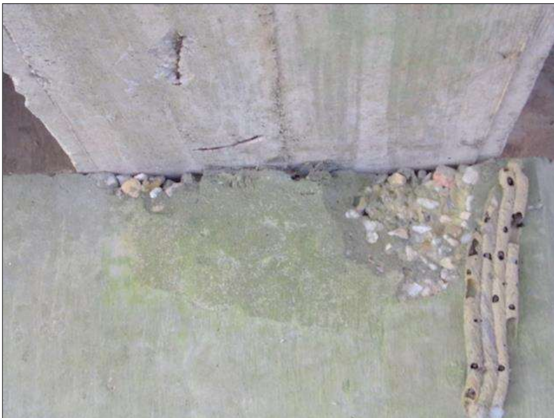
End Bent 2 Cap 1: (2) UP TO 8 INCHES X 6 INCHES X 1 INCHES DEEP SPALL ON WEST FACE OF BEAM 2 BLOCKOUT AT TOP OF CAP.
