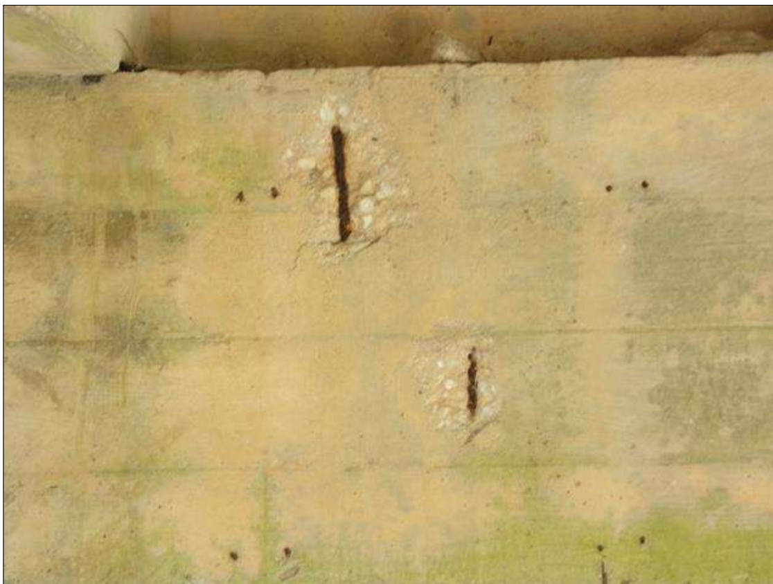
Bent 1 Cap 1: (2) UP TO 8 INCHES X 12 INCHES X 1/2 INCH DEEP SPALLS WITH EXPOSED REINFORCING ON WEST FACE BETWEEN BEAMS 2 AND 3.
