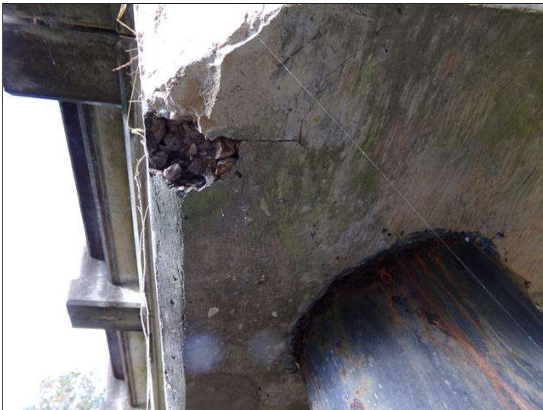
Bent 1 Cap 1: 4 INCH X 3 INCH X 1 INCH DEEP SPALL ON BOTTOM OF CAP AT SOUTH END
