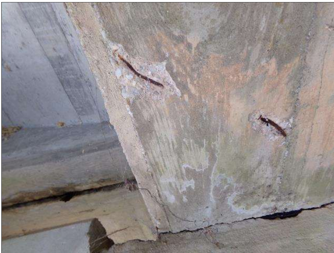
SPAN 2 Beam 4: (2) UP TO 3 INCHES X 2 1/2 INCHES X 1/2 INCH DEEP SPALL ON BOTTOM OF BEAM AT BENT 1
