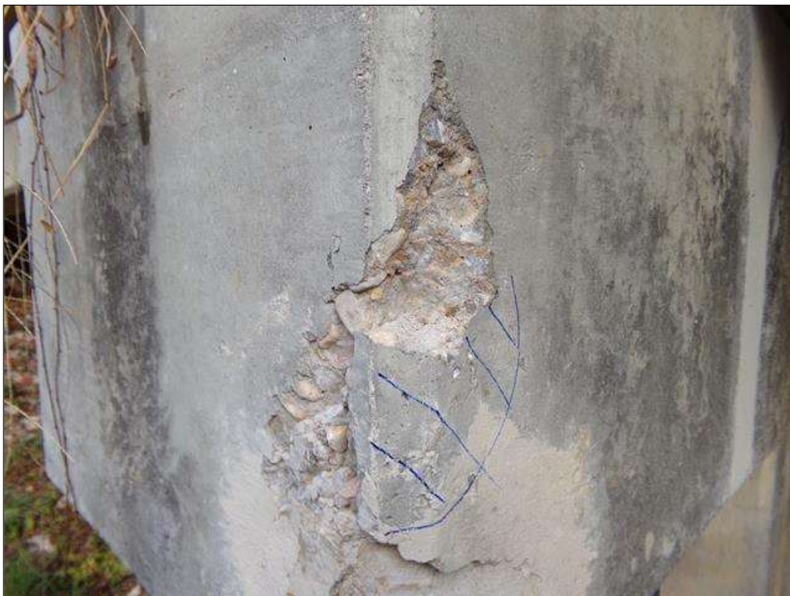
Bent 1 Cap 1: 10" X 10" X 1 1/2" DEEP SPALL AND AREA OF DELAMINATION AT SOUTHEAST CORNER
