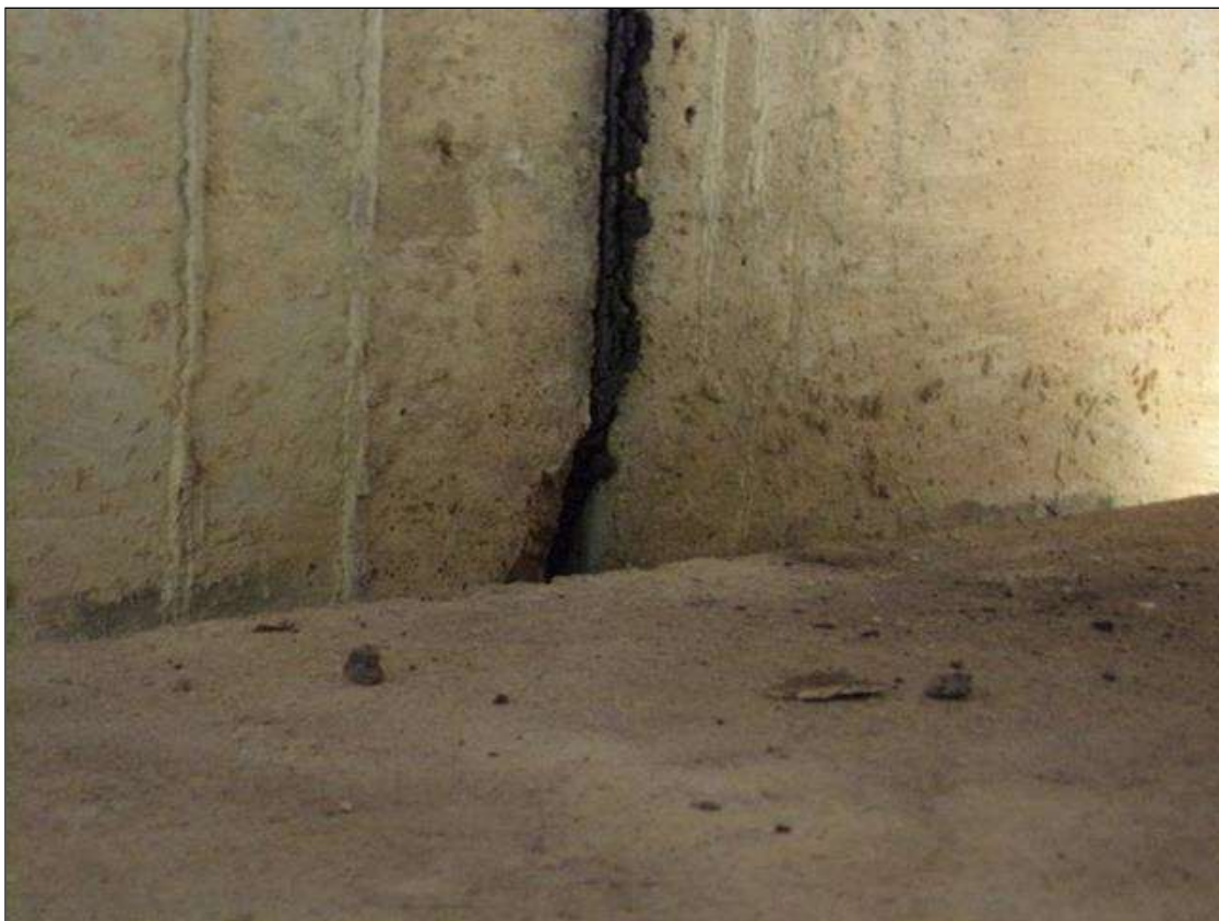
Span 2 Beam 1: 2 INCH X 4 INCH X 1 INCH DEEP SPALL ON LEFT SIDE OF BEAM AT BENT 1
