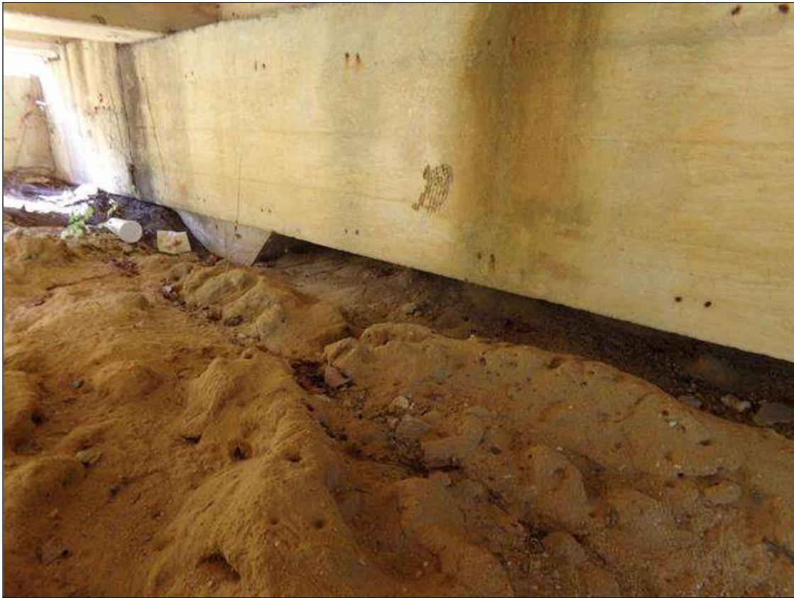
End Bent 1 Abutment: 29 FEET X 38 INCHES DEEP UNDERNEATH UNDER END BENT 1 CAP (PAR)
