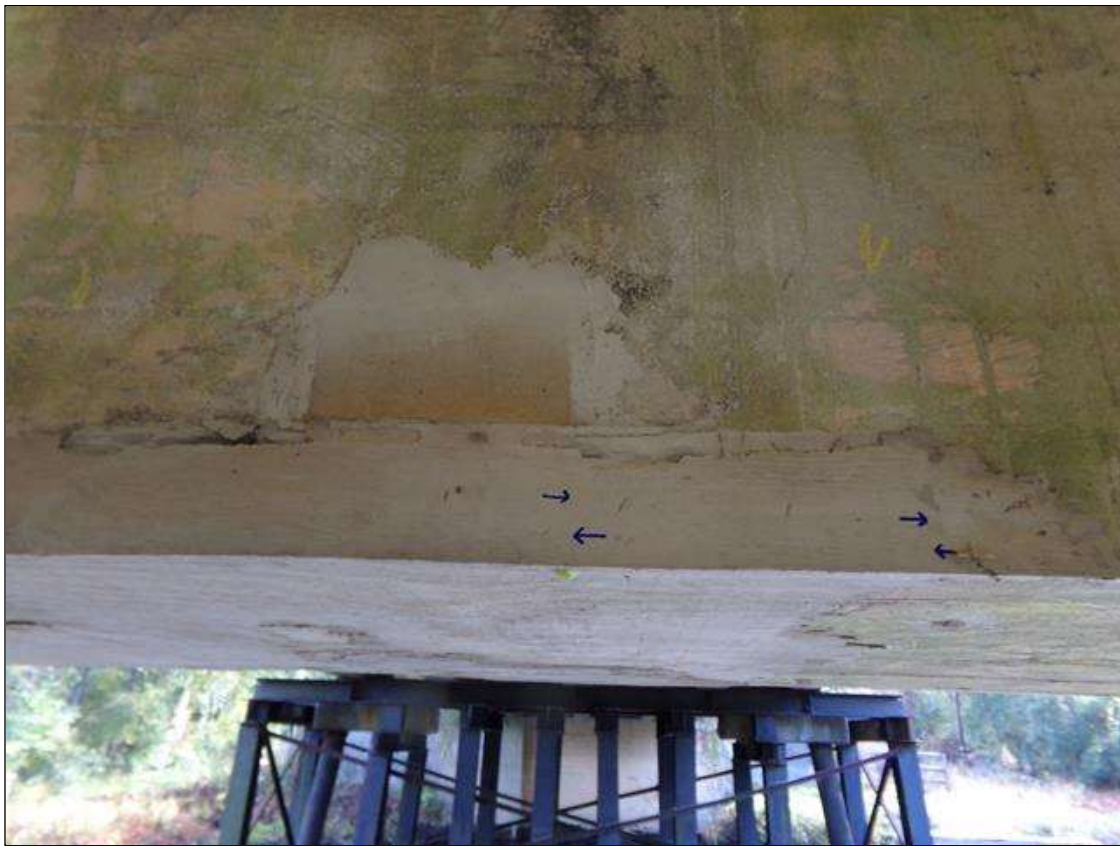
Bent 2 Cap 1: 21 INCHES X 4 INCHES X 3 INCHES DEEP SPALL WITH ASSOCIATED 32 INCHES X 1/32 INCHES VERTICAL CRACK ON WEST FACE BENEATH BEAM 3 AND ASSOCIATED 22 INCHES X 9 INCHES DELAMINATION ON BOTTOM FACE (PATCHED WITH HAIRLINE VERTICAL CRACKS)
