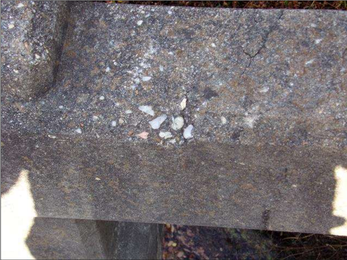
SPAN 4 Left Bridge Rail: 20 INCHES OF UP TO 1/2 INCHES GOUGES AND 1/16 INCHES WRAPAROUND CRACKS ON ALL FACES OF RAIL 15 FEET FROM BENT 3.
