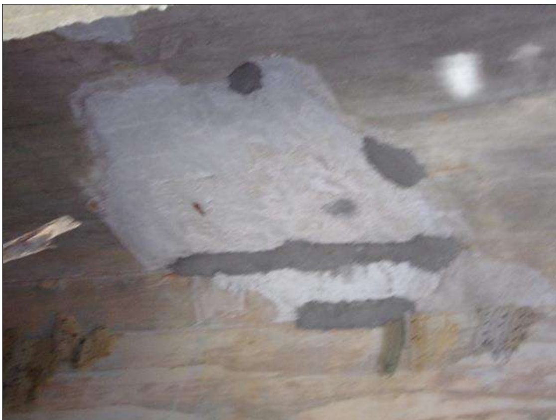
SPAN 4 Deck: 36 INCH X 24 INCH AREA OF PATCH WITH 2 INCH X 1 INCH X 1/2 INCH DEEP SPALL WITH EXPOSED REBAR ON BOTTOM OF DECK IN BAY 2 AT BENT 3
