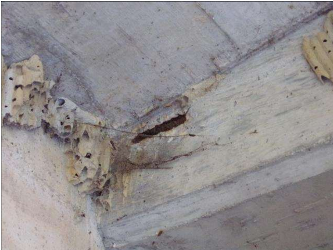
SPAN 3 Beam 1: 5 INCHES X 2 INCHES X 1/4 INCHES DEEP SPALL WITH EXPOSED REINFORCING ON WEST FACE OF BENT 2 END DIAPHRAGM BETWEEN BEAMS 1 AND 2.
