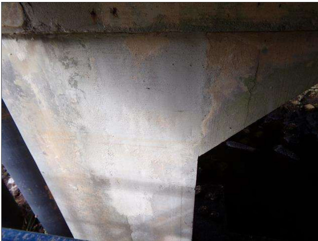
Bent 1 Pile 4: 18 INCHES X 46 INCHES SOUND PATCHED AREA ON EAST FACE AT TOP OF CAP.
