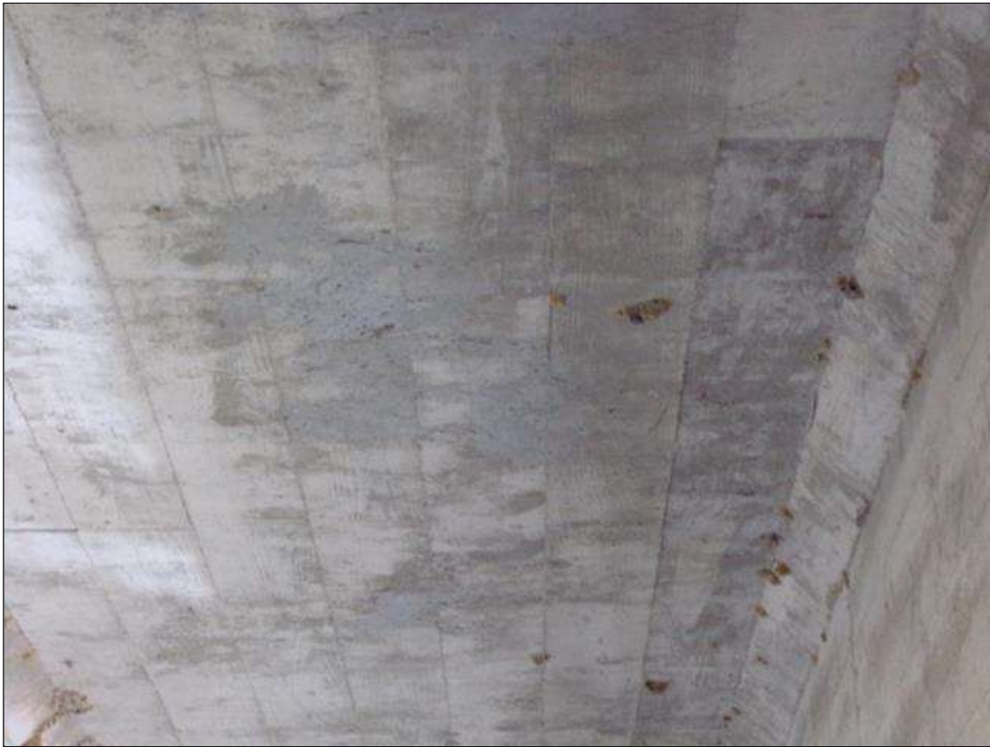
Span 2 Deck: 35 SQUARE FEET UP TO 2 FEET X 1 FEET PATCHED AREAS AT RANDOM THROUGHOUT DECK UNDERSIDE BETWEEN BEAMS 2 AND 4
