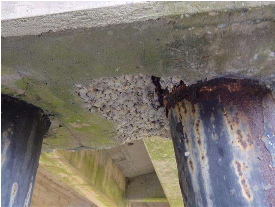
Bent 1 Cap 1: 14 INCHES X 26 INCHES X 2.5 INCHES DEEP SPALL ON BOTTOM FACE BETWEEN PILES 1 AND 2 (PAR)
