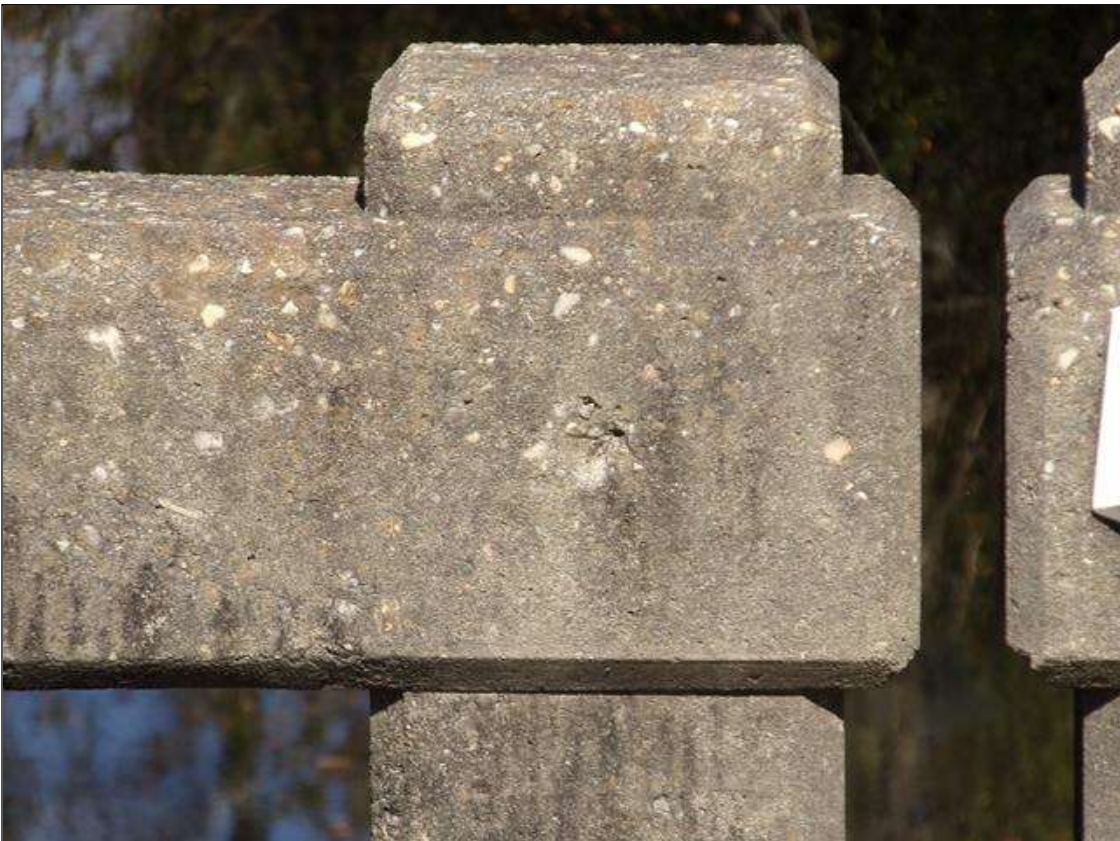
SPAN 4 Left Bridge Rail: 3 INCHES X 2 INCHES X 2 INCHES DEEP SPALL ON TOP AND SOUTH FACES, 19 FEET FROM END BENT 2.
