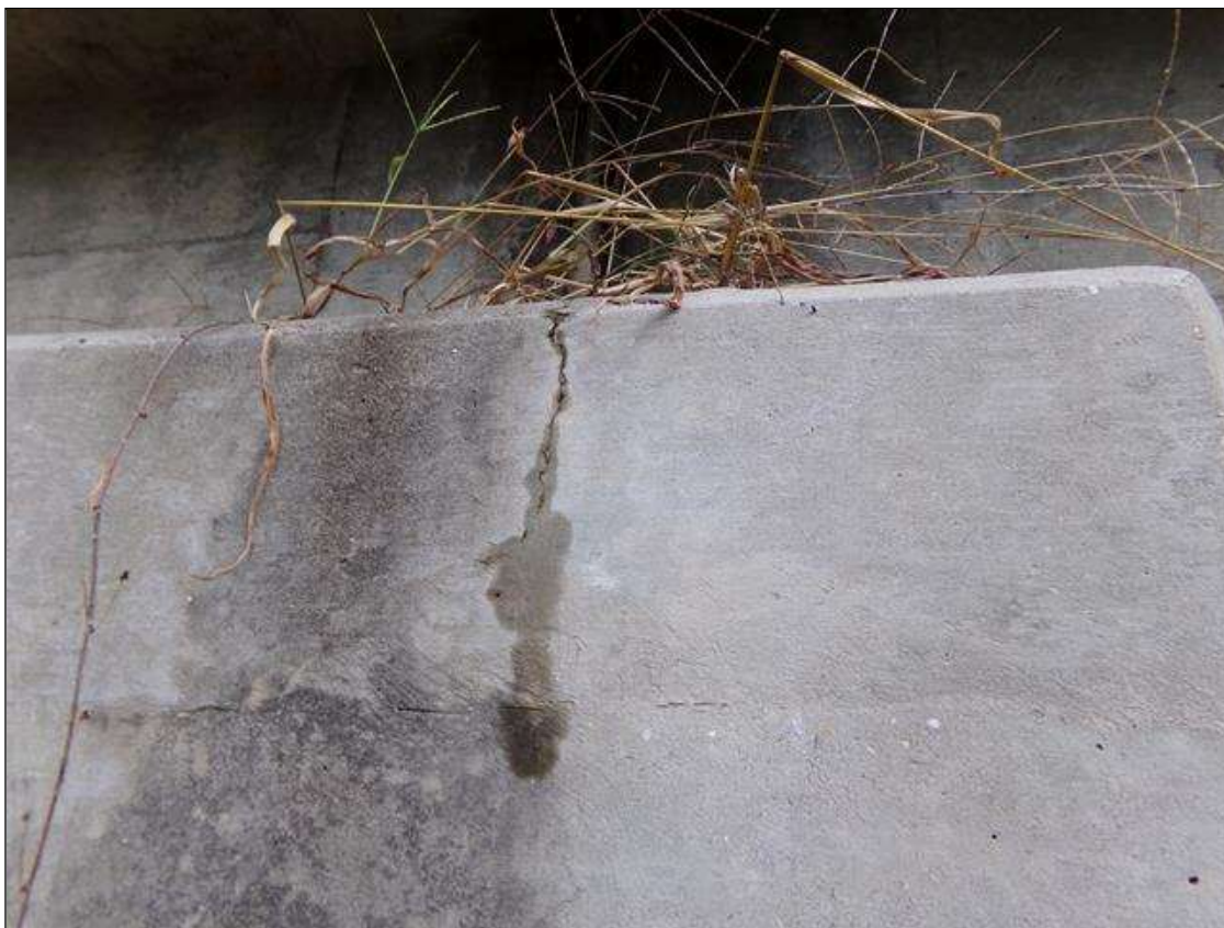
Bent 1 Cap 1: 9 INCHES X 1/32 INCHES VETICAL CRACK ON SOUTH FACE AT TOP OF CAP
