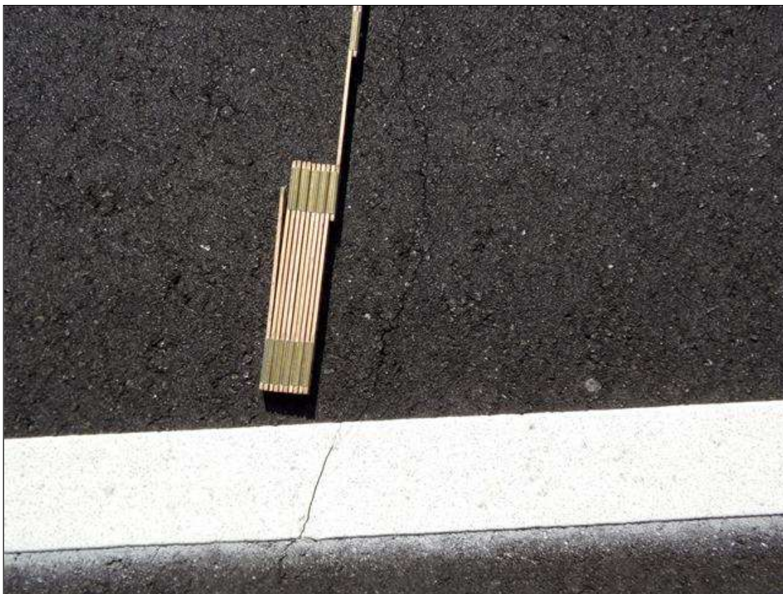
Span 4 Wearing Surface: 6 SQUARE FEET HAIRLINE TRANSVERSE CRACK AT END BENT 2
