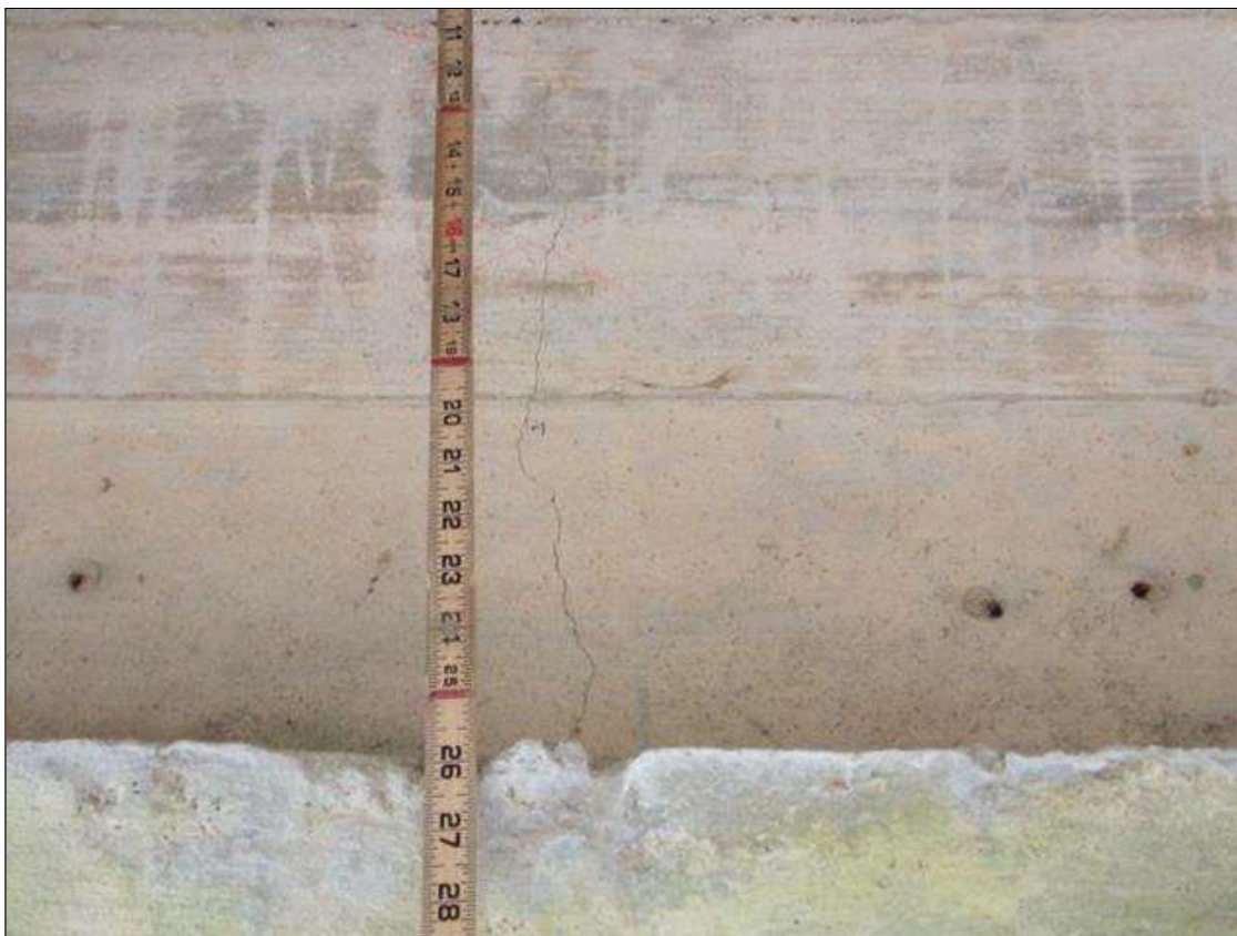
SPAN 2 Beam 2: 26 INCHES X 1/64 INCHES VERTICAL CRACK ON EAST FACE OF BENT 1 END DIAPHRAGM BETWEEN BEAMS 2 AND 3 BEGINNING AT TOP OF CAP.
