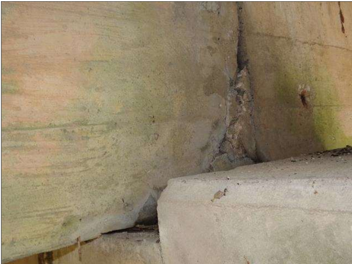
SPAN 2 Beam 4: 9 INCHES X 4 INCHES X 1/2 DEEP INCHES SPALL WITH ASSOCIATED 18 INCHES X 9 INCHES DELAMINATION ON SOUTH FACE AT BENT 2.
