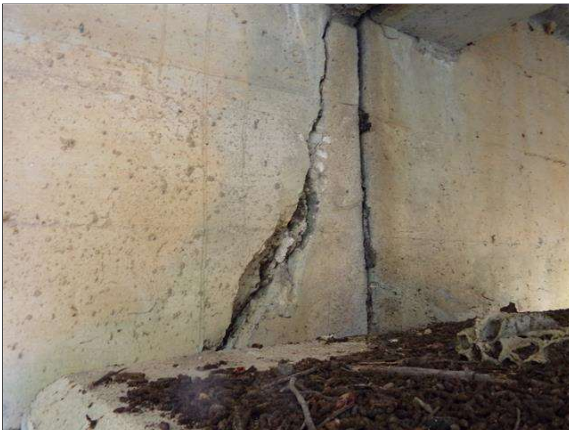
SPAN 3 Beam 2: 9 INCHES X 20 INCHES X 2 INCHES DEEP SPALL ON NORTH FACE AT BENT 2
