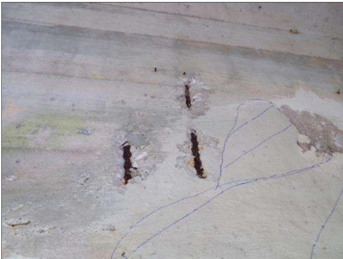
SPAN 2 Beam 2: (4) UP TO 4 INCH X 6 INCH X 1/2 INCH DEEP SPALLS WITH EXPOSED REINFORCING ON EAST FACE, 3 FEET FROM BENT 2.
