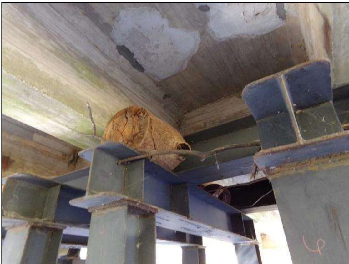
3 FEET X 4 FEET X 18 INCHES HIGH DRIFT AND DEBRIS ON SPAN 4 FACE OF CRUTCH BENT ON TOP OF PILE 4 (SPAN 3 FACE SIMILAR)
