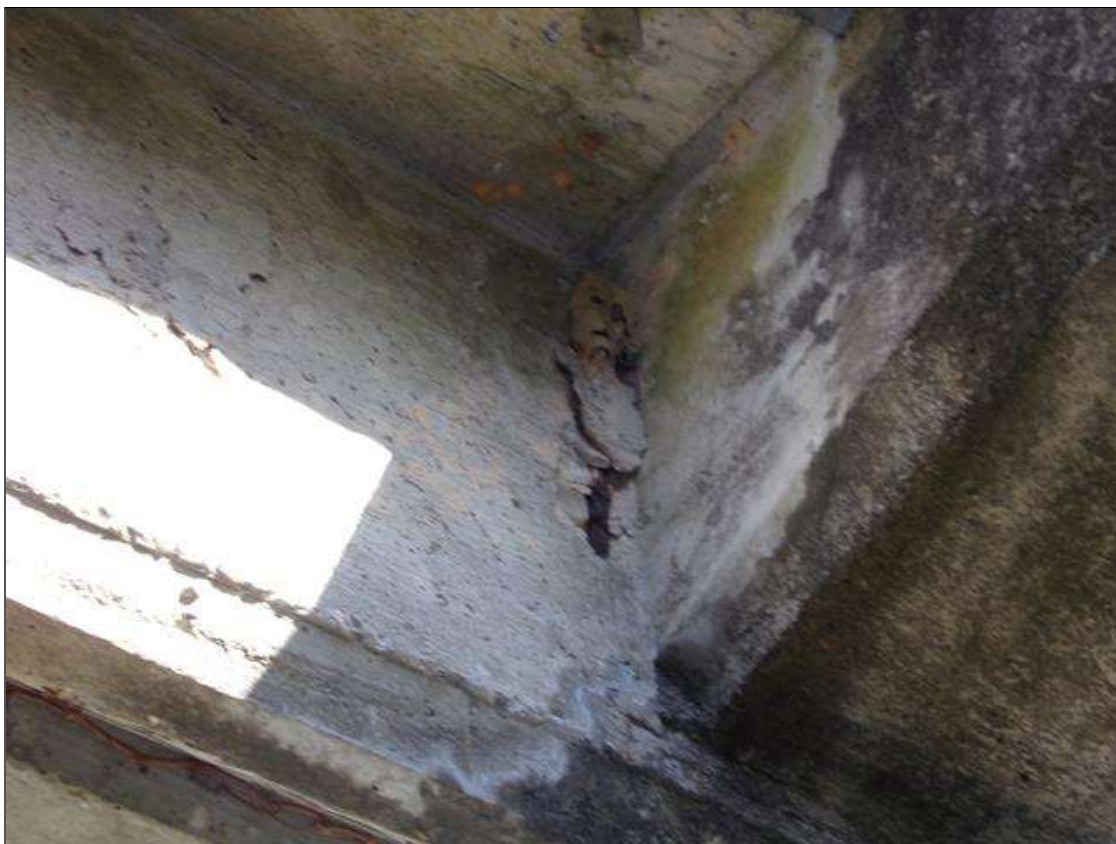
Span 4 Deck: 4 INCHES X 8 INCHES X 3/4 DEEP INCHES SPALL WITH EXPOSED REINFORCING AND AREA OF DELAMINATION ON SOUTH FACE AT WEST FACE OF 3RD RAIL POST BLOCKOUT FROM END BENT 2.
