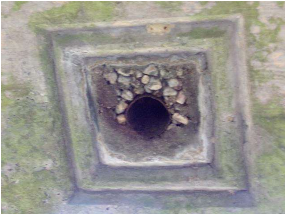
SPAN 2 Deck: 5 SQUARE FEET OF HONEYCOMBING AT RANDOM THROUGHOUT DRAINAGE OUTLETS ON THE NORTH OVERHANG
