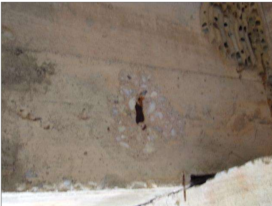
SPAN 2 Beam 4: 6 INCHES DIAMETER X 1/2 INCH DEEP SPALL WITH EXPOSED REINFORCING ON NORTH FACE AT BENT 1.
