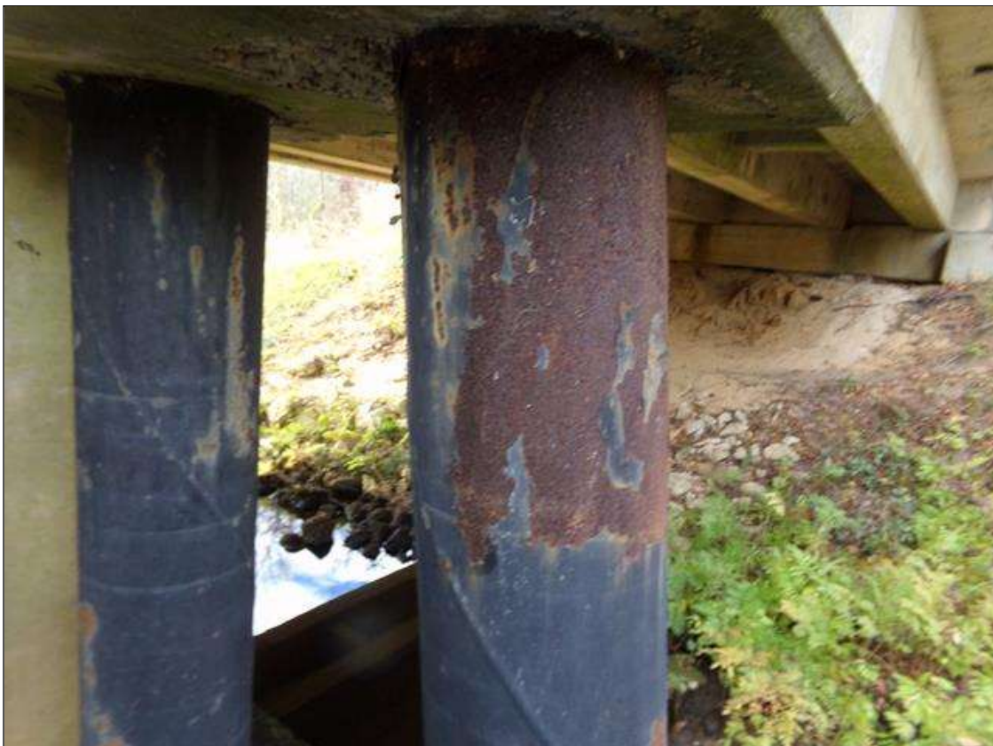
Bent 1 Pile 1: 7 FEET OF PEELING PAINT WITH RUST AND SURFACE RUST AT RANDOM THROUGHOUT
