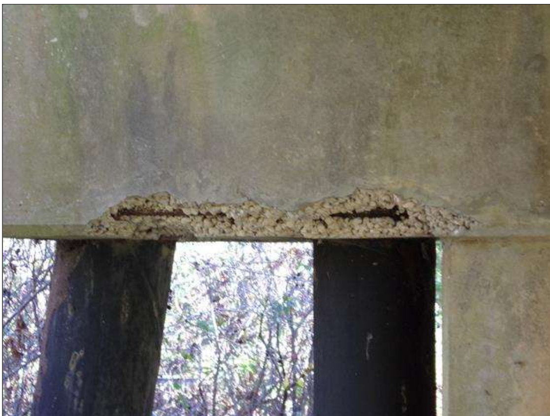
Bent 1 Cap 1: 45 INCHES X 7 INCHES X 6 INCHES DEEP SPALL WITH EXPOSED REINFORCING ON WEST FACE BENEATH BEAM 1 AT BOTTOM OF CAP (PAR)
