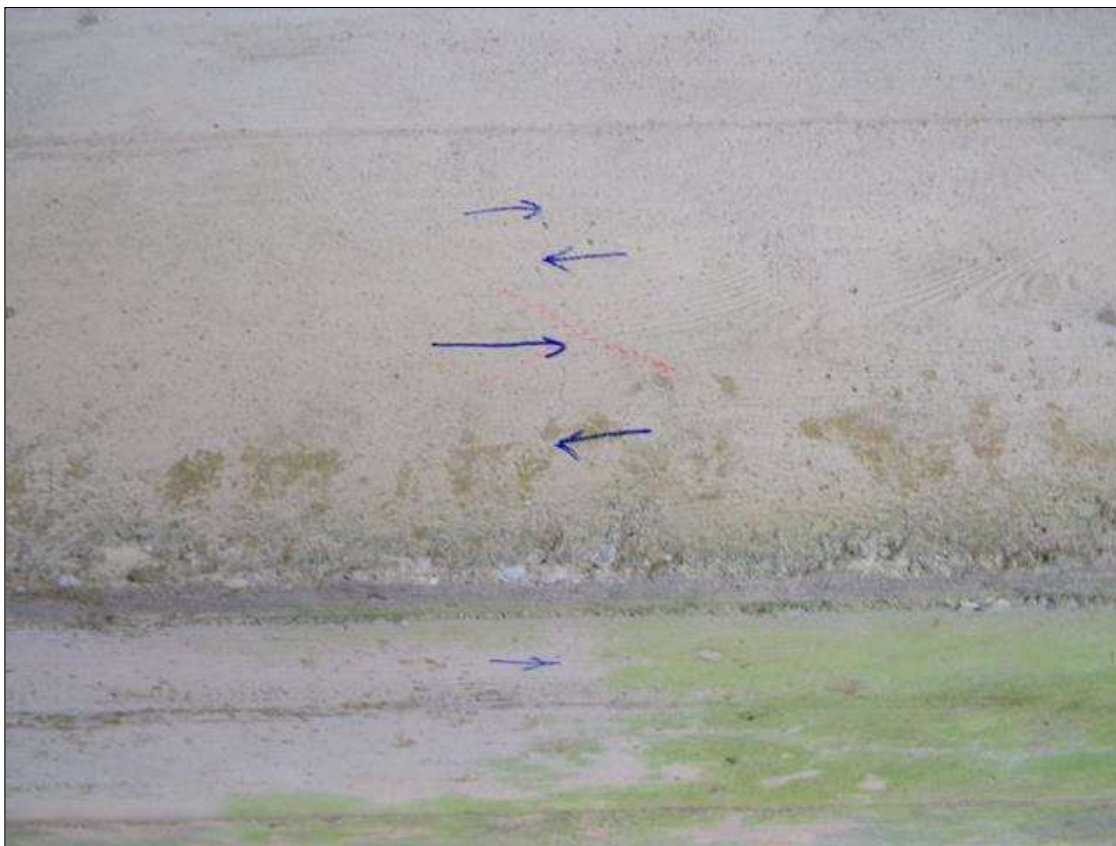
Span 2 Beam 2: (13) UP TO 1/64 INCHES WRAPAROUND CRACKS AT RANDOM THROUGHOUT.
