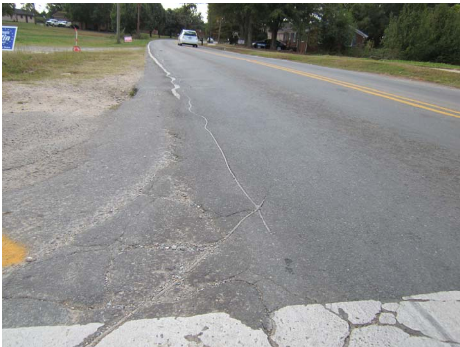
Exhibit A-19: Photograph of Moderate Rutting and Alligator Cracking (Edge) along Potter Road near the Intersection
