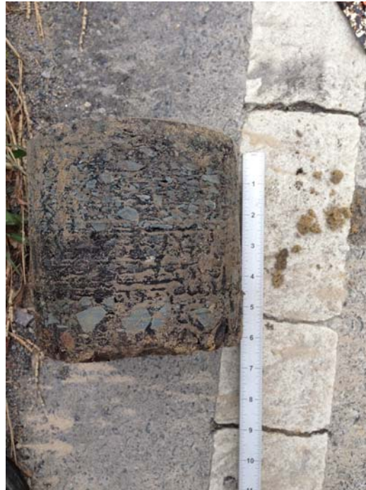
Exhibit A-20: Photograph of pavement core HA-01. Core HA-02 similar in condition and thickness.
