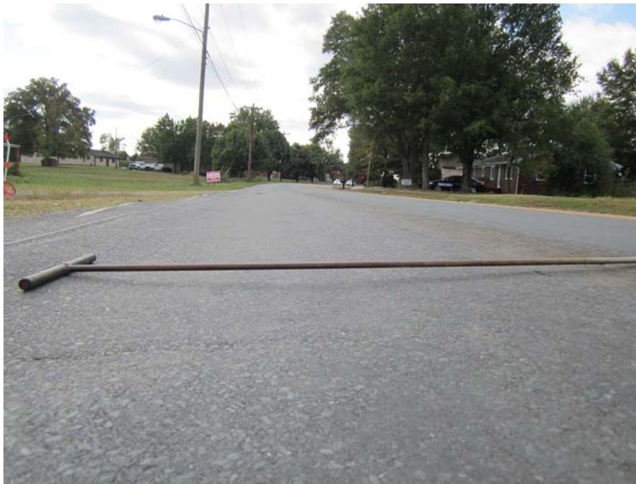
Exhibit A-17: Photograph of Moderate Rutting along Potter Road south of the Intersection
