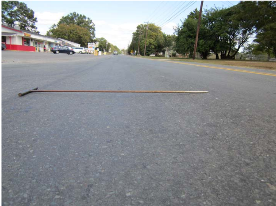
Exhibit A-18: Photograph of Moderate Rutting along Potter Road north of the Intersection
