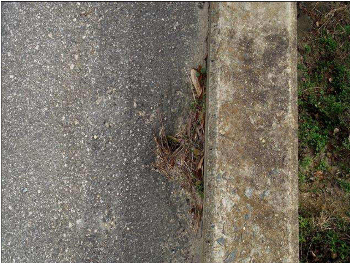
DRAINS CLOGGED ALONG THE RIGHT SIDE CURBLINE- LEFT SIDE SIMILAR
