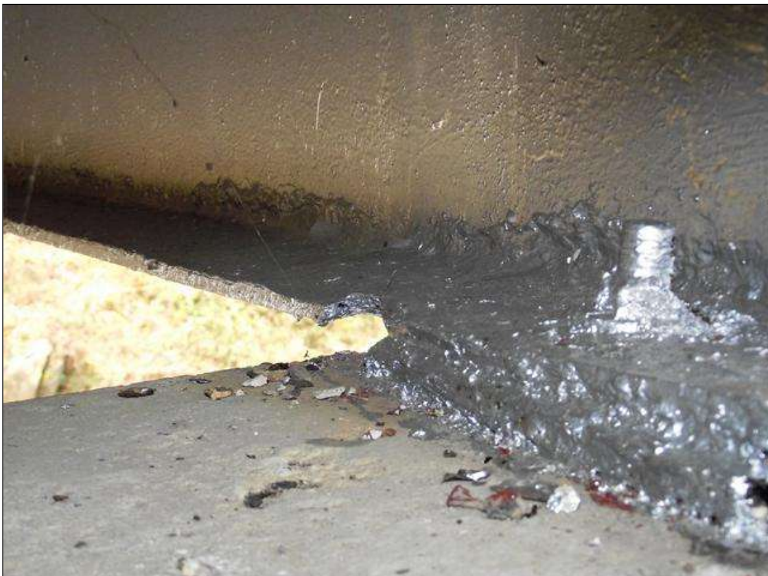
SECTION LOSS IN THE RIGHT SIDE BOTTOM FLANGE OF BEAM 1 IN SPAN 2 OVER BENT 1
