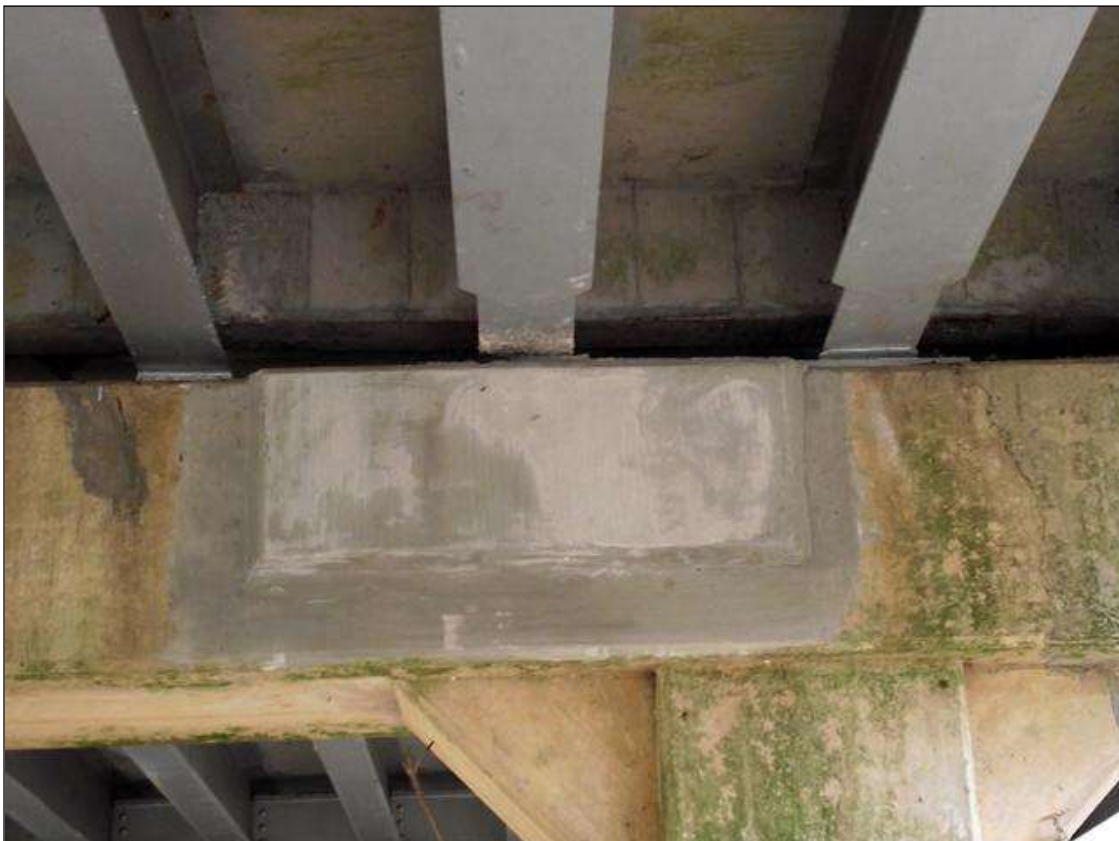
SPALL WITH EXPOSED REBAR IN FACE OF CAP AT BENT 3 SPAN 3 SIDE UNDER BAY 9 REPAIRED
