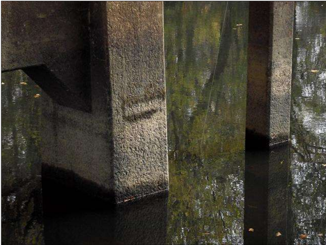
WATER ABRASION WITH EXPOSED AGGREGATE IN THE FLOWZONE OF BENT COLUMNS
