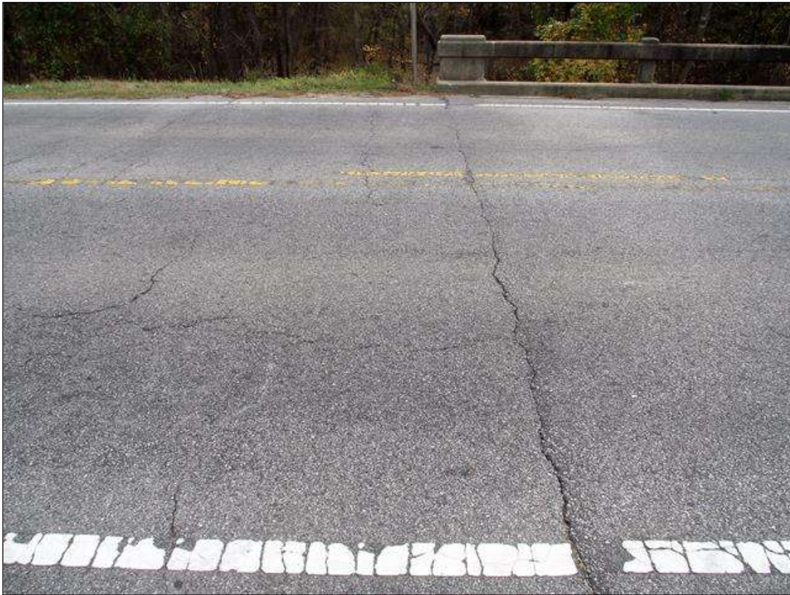
TRANSVERSE CRACK IN WEARING SURFACE OVER END BENT 2 AND IN APPROACH 2
