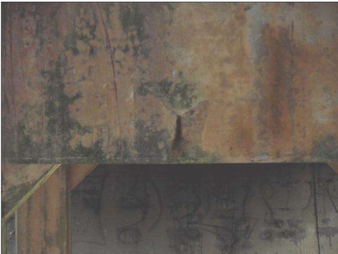
SPALL WITH EXPOSED REBAR IN FACE OF CAP AT BENT 1 SPAN 1 UNDER BAY 6
