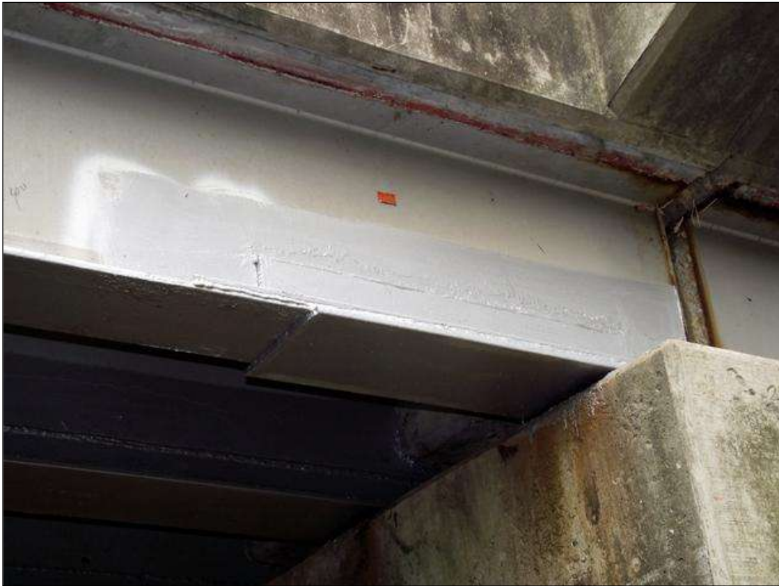
PLATE REPAIR AT THE END OF BEAM 13 OVER BENT 3 SPAN 3 SIDE - OTHER REPAIRS SIMILAR THROUGHOUT STRUCTURE
