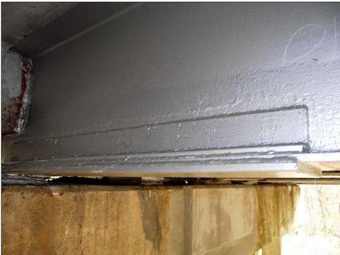
PLATE REPAIR DETAIL FOR BEAM 7 OVER BENT 3 SPAN 3 SIDE - OTHER REPAIRS SIMILAR AT THIS BENT
