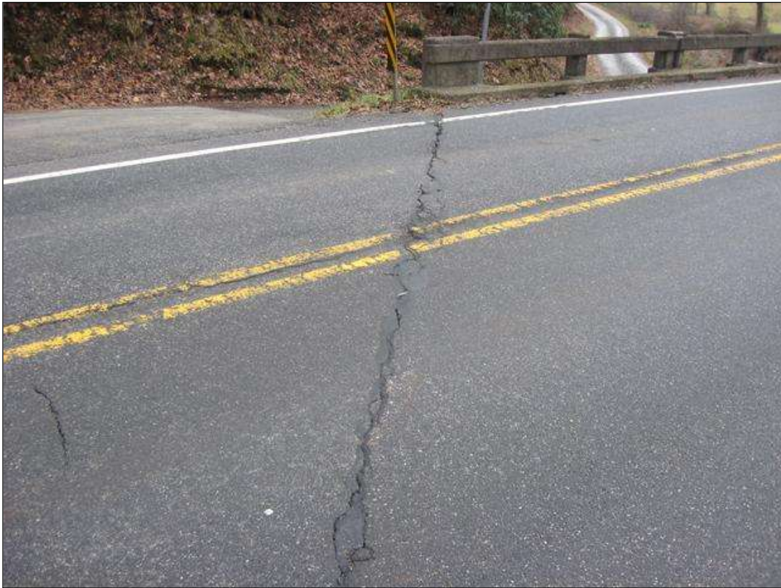
CRACK IN ASPHALT WEARING SURFACE ABOVE END BENT 2.
