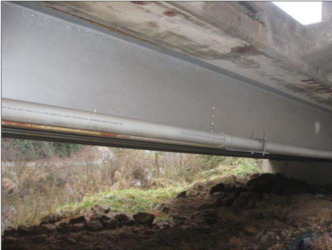
UTILITY ON DOWNSTREAM SIDE.
