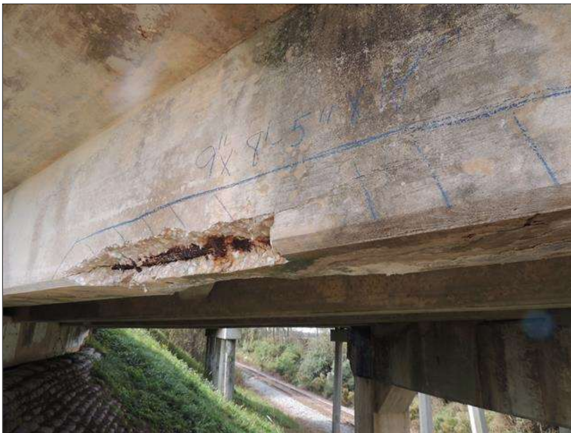
Span 1 Beam 4: 9 Feet of Delamination/Spall/Patched Area: Spall greater than 1 in. deep or greater than 6 in. diameter. Patched area that is unsound or showing distress. Does not warrant structural review. SPAN 1 G4 CRACKED AND DELAMINATED SPALL AREA AT MID SPAN ALONG LEFT AND RIGHT SIDE AND UNDER BOTTOM 9" UP FACE 8' 5" LONG 18" WIDE.
