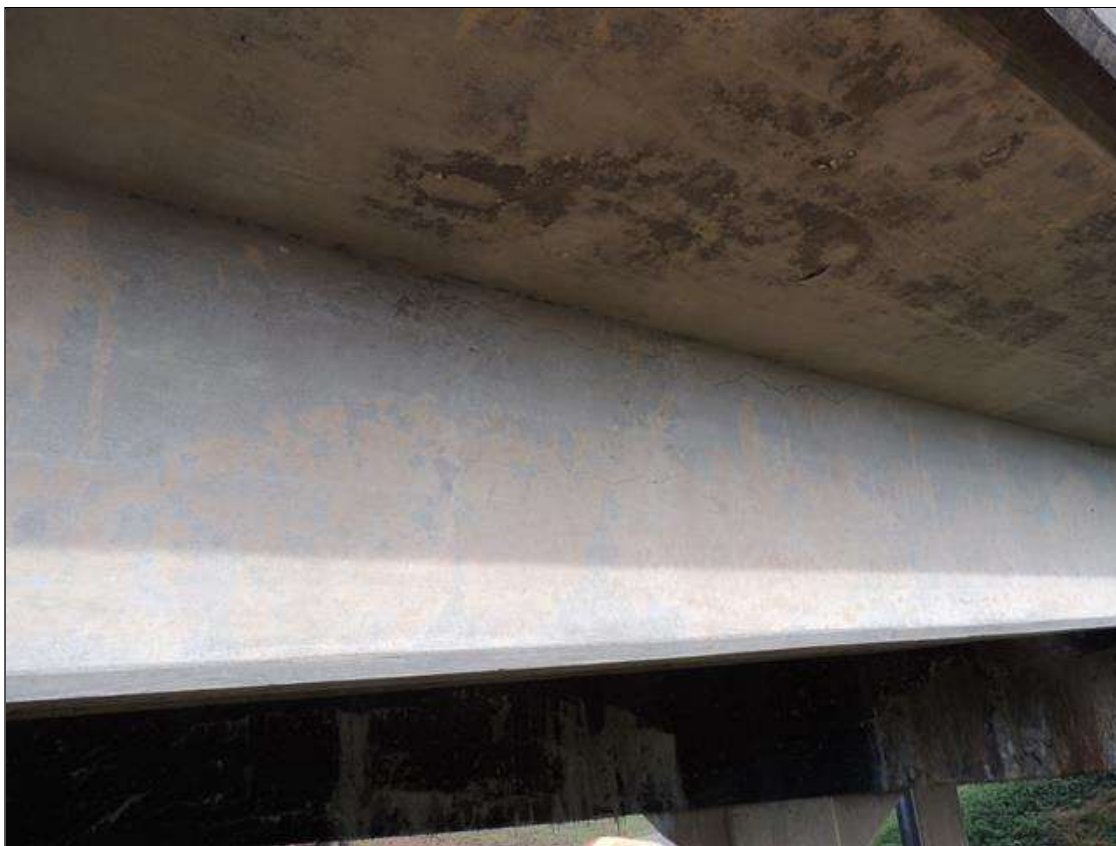
Span 4 Beam 1: 30 Feet of Cracking (RC and Other): Width 0.012-0.05 in. or spacing of 1.0-3.0 ft. LEFT SIDE OF G 1 SCATTERED MAP CRACKING FROM BENT 3 TO BENT 4.
