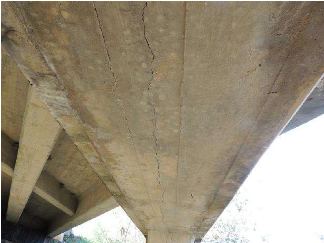
Bent 4 Cap : 10 Feet of Cracking (RC and Other): Width greater than 0.05 in. or spacing of less than 1 ft. BOTTOM OF CAO HAS SCATTERED CRACKING FROM COL. 2 TO COL. 3.
