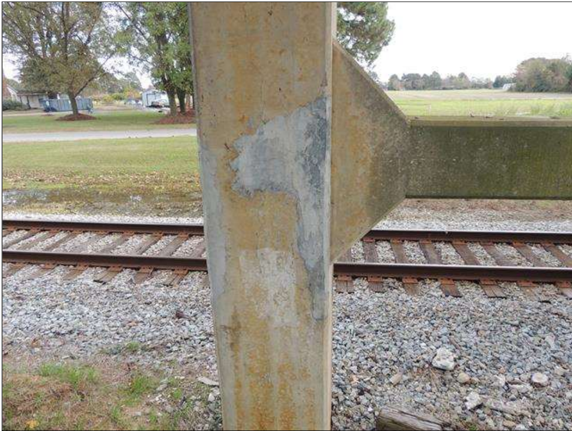
BENT 3 COL. 3 NORTH FACE HAS 2 PATCHED AREAS 4' ABOVE GROUND EXTENDING & 30 " WIDE.
