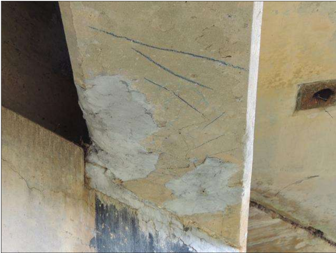
Span 2 Beam 1: 4 Feet of Delamination/Spall/Patched Area: Delaminated. Spall 1 in. or less deep or 6 in. or less in diameter. Patched area that is sound. SPAN 2 LEFT AND RIGHT SIDE AND BOTTOM OF G1 CRACKED AND DELAMINATED AREAS 18" WIDE FROM BENT 1 CAP OUT 4' AND 4" UP FACE.
