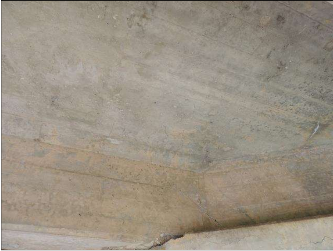
Span 2 Deck: 40 Square Feet of Delamination/Spall: Delaminated. Spall 1 in. or less deep or 6 in. or less in diameter. SPAN 2 BOTTOM OF DECK IN BAY 1 CRACKED AND DELAMINATED FROM BENT OUT 10' 4' WIDE.
