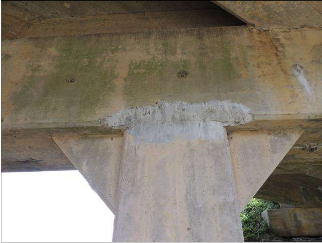
Bent 1 Cap : 0 Feet of Delamination/Spall/Patched Area: Delaminated. Spall 1 inch or less deep or 6 inches or less in diameter. Patched area that is sound BENT 1 NORTH FACE OF CAP PATCHED AREA ALONG BOTTOM EDGE AT COL 2 5" UP FACE 45" LONG.
