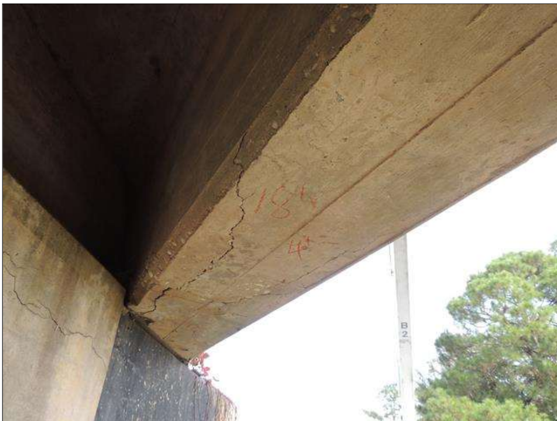
Span 1 Beam 4: 4 Feet of Delamination/Spall/Patched Area: Delaminated. Spall 1 in. or less deep or 6 in. or less in diameter. Patched area that is sound. SPAN 1 LEFT AND RIGHT SIDE AND BOTTOM OF G4 AT BENT 1 IS CRACKED AND DELAMINATED 6" UP EACH FACE 18" WIDE UNDER BOTTOM 4' LONG.
