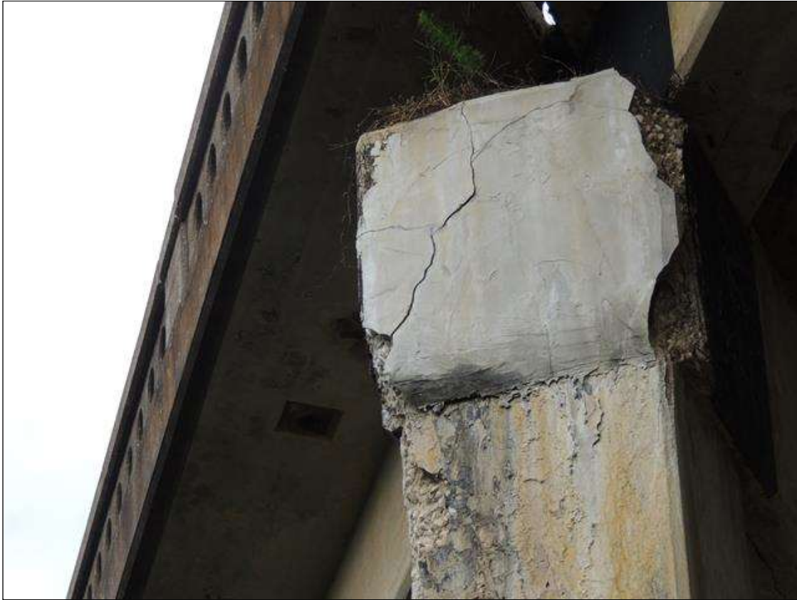
Bent 3 Cap : 12 Feet of Delamination/Spall/Patched Area: The condition warrants structural review to determine the effect on strength and serviceability of the element or the bridge; OR a structural review has been completed and the defects impact strength or serviceability of the element or bridge. LEFT END OF CAP IS CRACKED, SPALLED DELAMINATED AND DETERIORATED 37" X 37". 3' X 5" DEEP ON NORTH AND SOUTH FACES.
