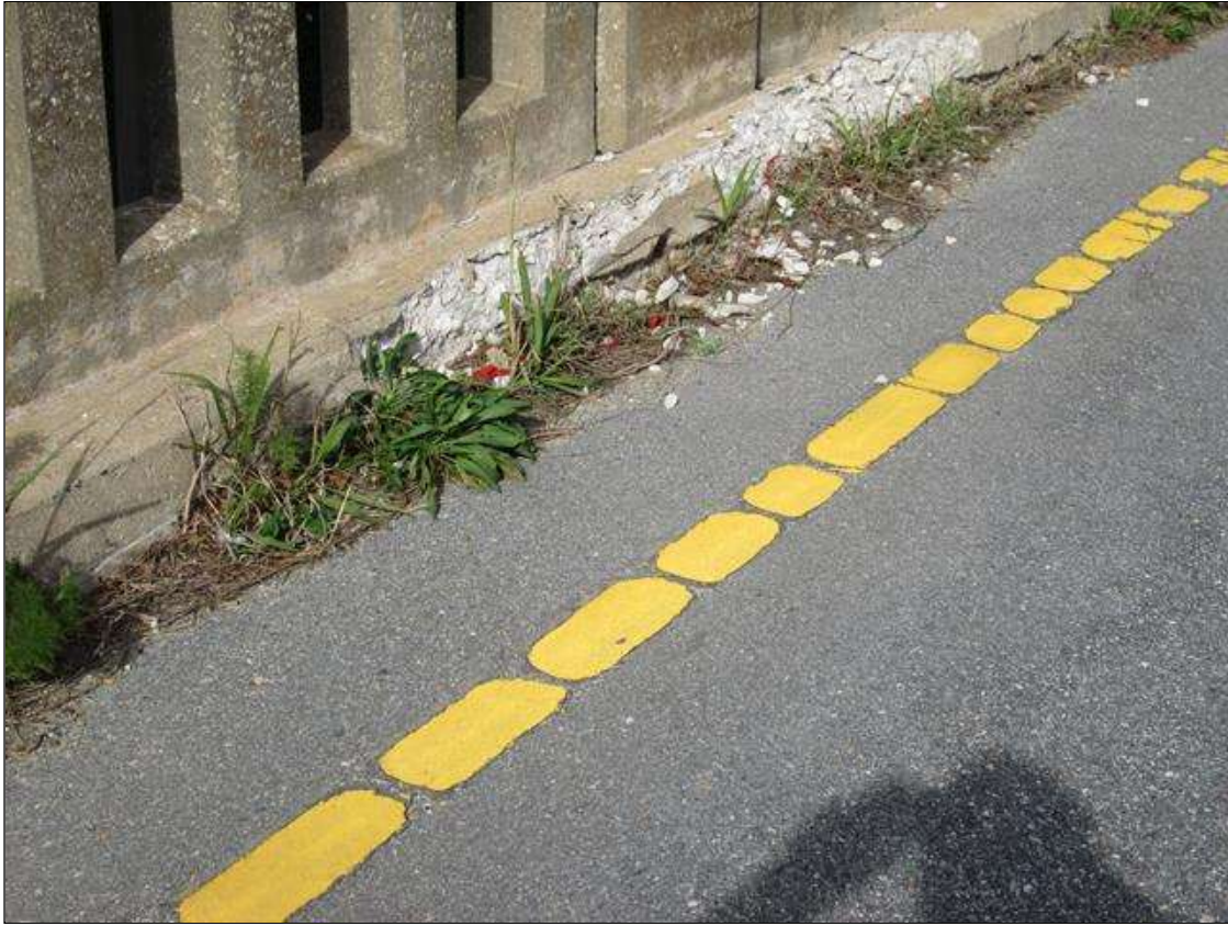
Span 1 Right Bridge Rail: 10 Feet of Delamination/Spall/Patched Area: Delaminated. Spall 1 in. or less deep or 6 in. or less in diameter. Patched area that is sound. LEFT CURB 10' FROM END BENT 1 IS SPALLED , CRACKED AND DELAMINATED. AREA IS 10' LONG 10" HIGH AND 8" BACK ON TOP
