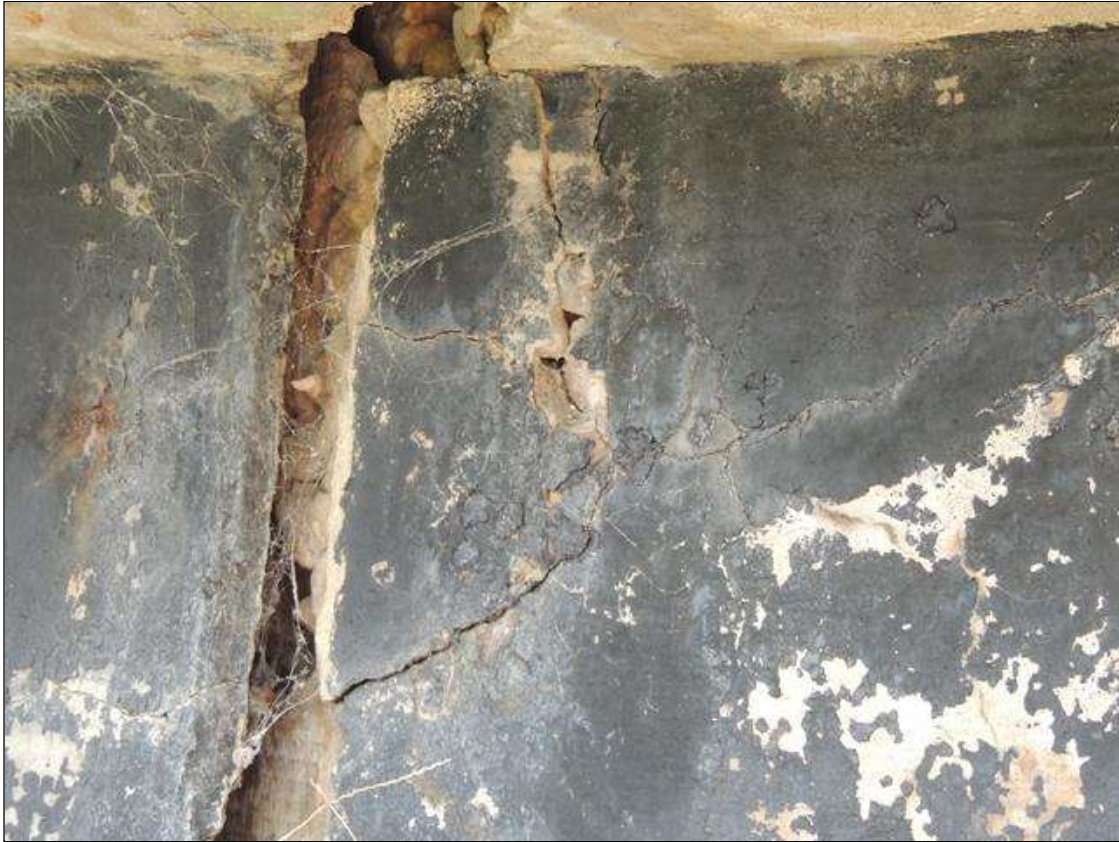
Span 2 Beam 1: 1 Feet of Delamination/Spall/Patched Area: Delaminated. Spall 1 in. or less deep or 6 in. or less in diameter. Patched area that is sound. SPAN 2 LEFT SIDE OF G1 OVER BENT 2 7" X 7" CRACK AREA OVER TOP OF GIRDER.
