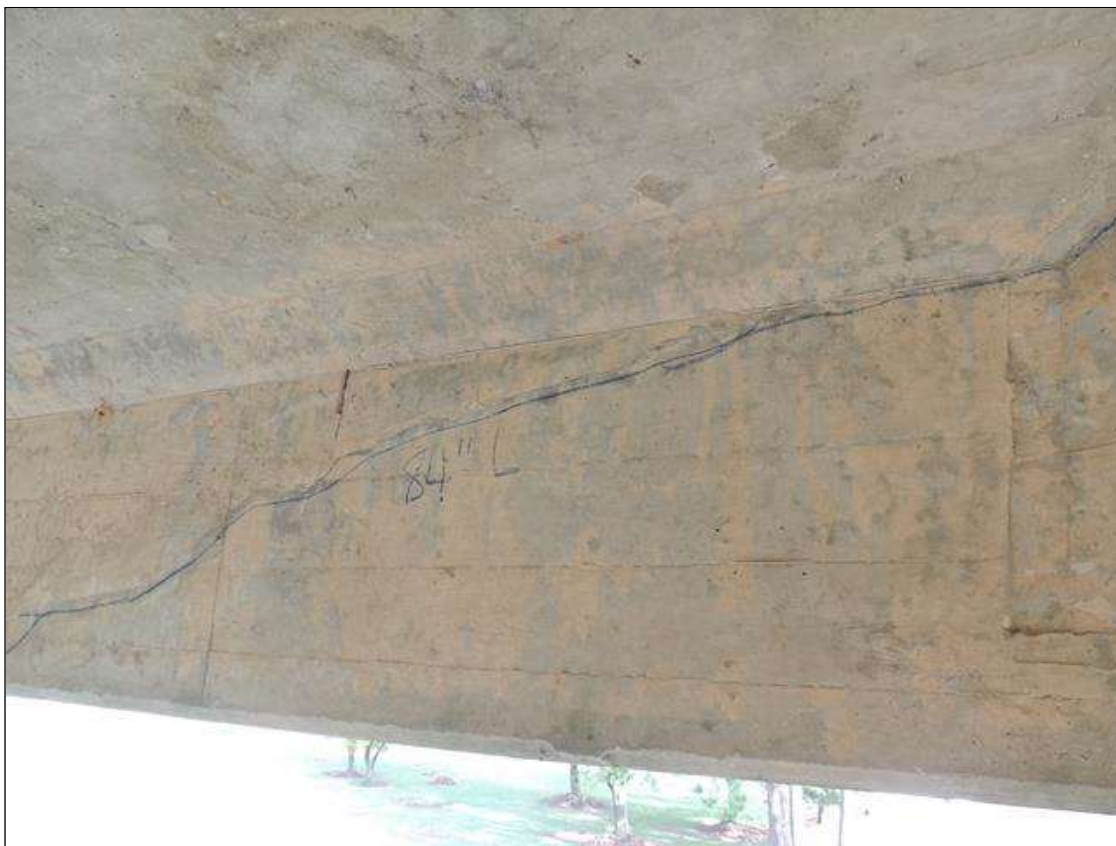
Span 2 Beam 4: 7 Feet of Cracking (RC and Other): Width 0.012-0.05 in. or spacing of 1.0-3.0 ft. SPAN 2 LEFT SIDE OF G4 HAS A DIAG CRACK COMING OFF THE INTERIOR DIAPHRAGM 7' LONG FROM TOP TO BOTTOM.
