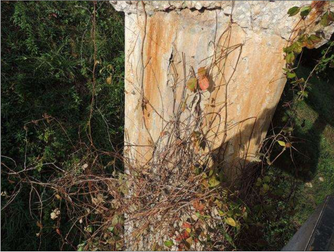
Bent 4 Pile 1: 0 Each of Delamination/Spall/Patched Area: Spall greater than 1 in. deep or greater than 6 in. diameter. WEST FACE OF COL. HAS CRACKS WITH HEAVY EFFLO STAINS FROM TOP DOWN 14' 30" WIDE.
