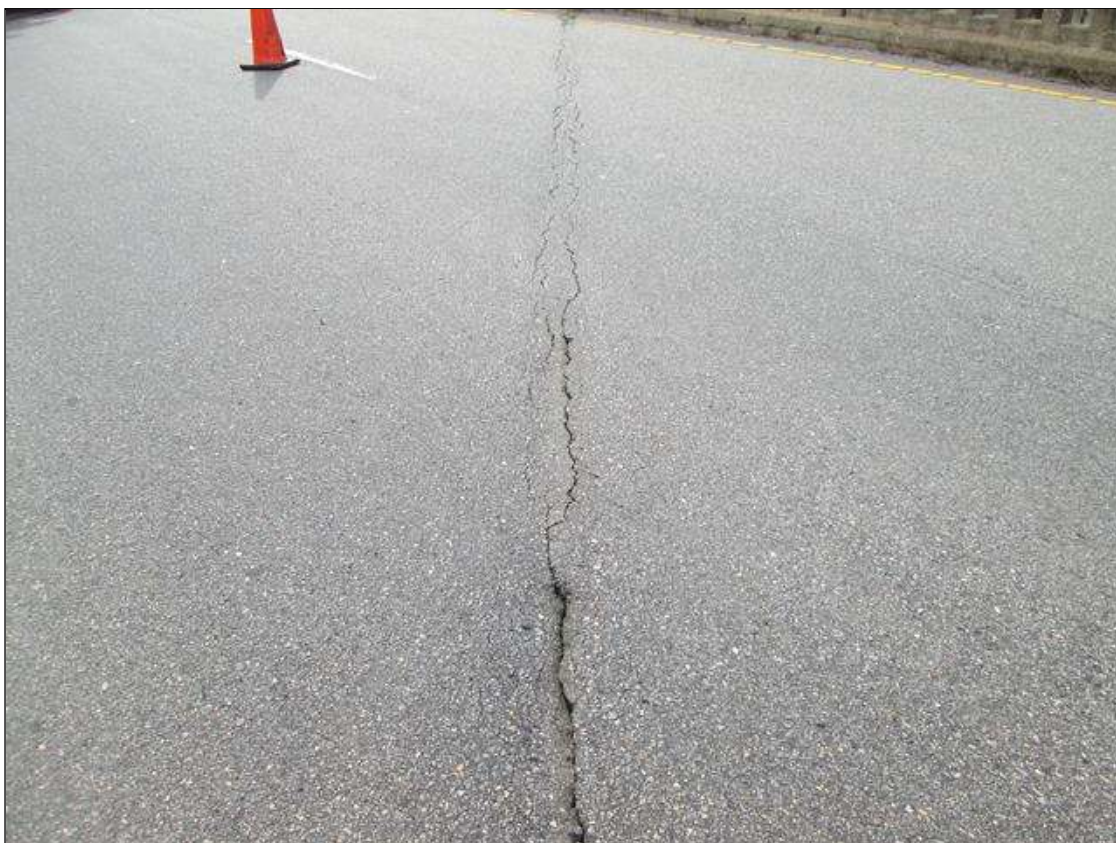
Expansion Joint 5 : 32 Feet of Seal Cracking: Surface crack. ASPHALT OVER BENT 4 IS CRACKED IN BOTH LANES FROM LEFT CURB OUT 32'.
