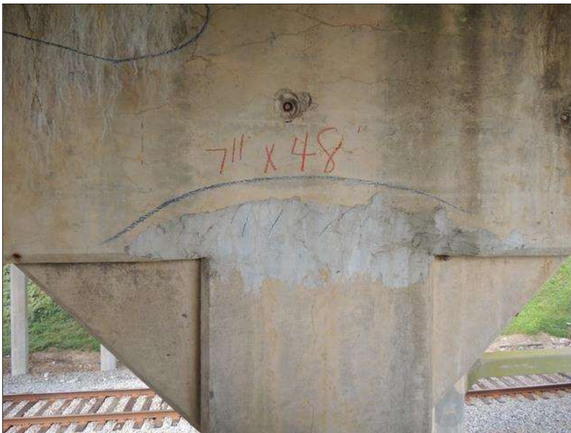
Bent 1 Cap : 4 Feet of Delamination/Spall/Patched Area: Delaminated. Spall 1 inch or less deep or 6 inches or less in diameter. Patched area that is sound BENT 1 SOUTH FACE OF CAP PATCHED AREA ALONG THE BOTTOM EDGE AT COL 2 7" UP FACE AND 40" LONG.
