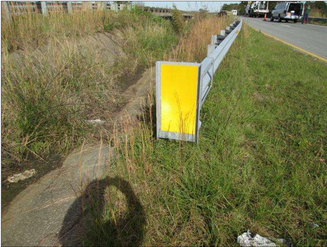
GUARDRAIL TERMINAL END
