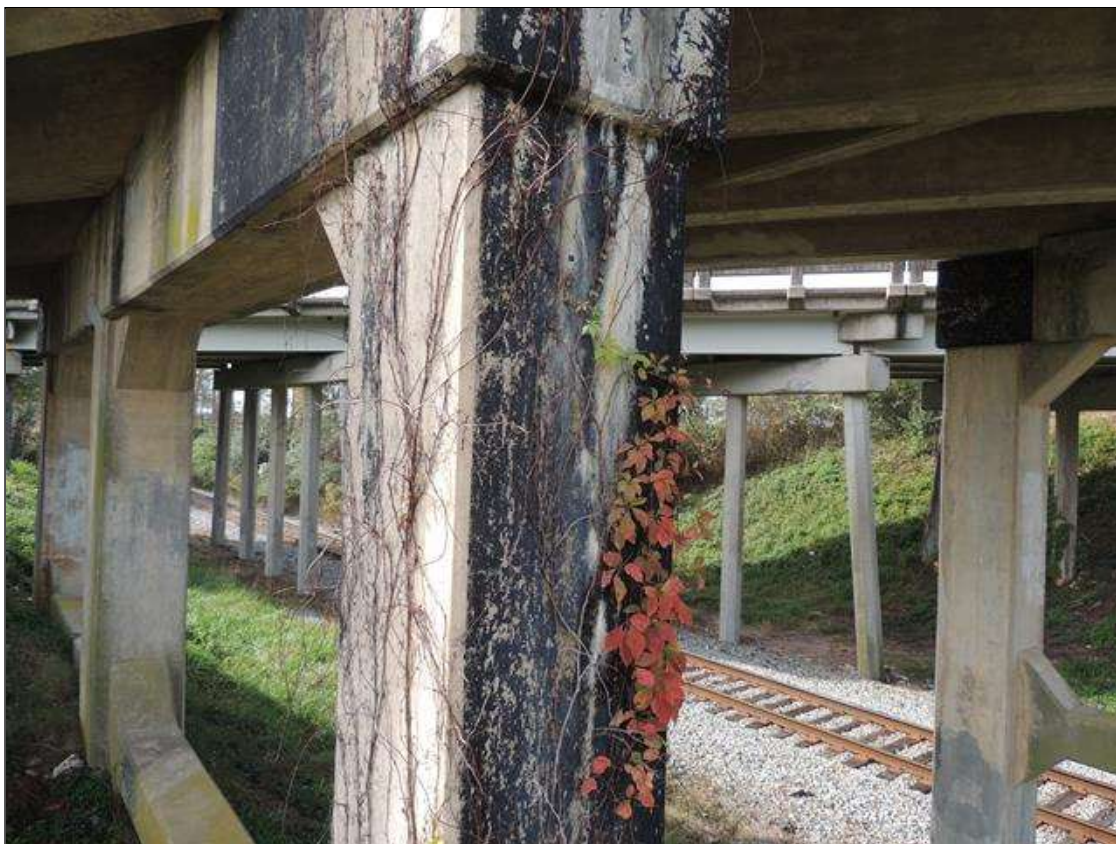
Bent 1 Pile 3: 1 Each of Delamination/Spall/Patched Area: Delaminated. Spall 1 in. or less deep or 6 in. or less in diameter. Patched area that is sound. BENT 1 EAST FACE OF COL 3 CRACKED AND DELAMINATED WITH EFFLO STAINS TO- DOWN 12'
