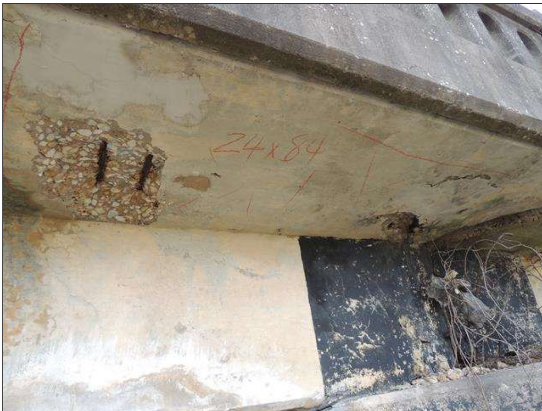
Span 4 Deck: 14 Square Feet of Exposed Rebar: Present without measurable section loss. BOTTOM OF DECK RIGHT OVER HANG HAS 2 SPALL AND DELAMINATED AREAS WITH REBAR EXPOSED NEAR BENT 4. AREAS ARE 16" X 20" X 2" & 23" X 26" X 2".
