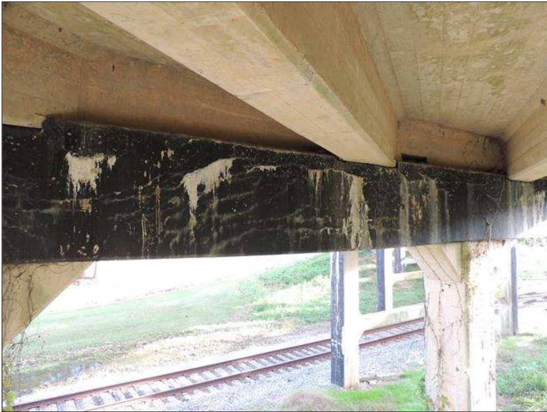
Bent 4 Cap : 6 Feet of Cracking (RC and Other): Width greater than 0.05 in. or spacing of less than 1 ft. NORTH FACE OF CAP HAS SCATTERED MAP, HORIZONTAL AND VERTICAL CRACKS.
