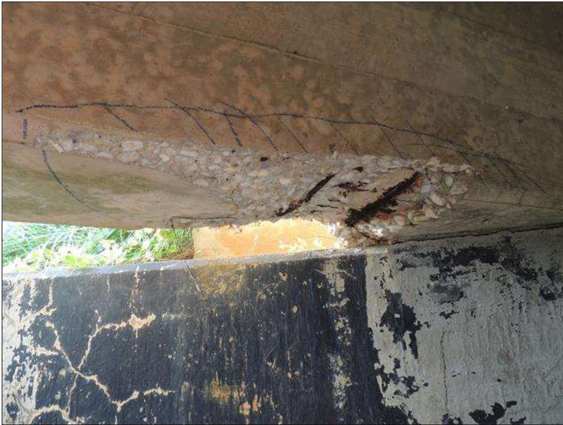
Span 5 Beam 1: 3 Feet of Delamination/Spall/Patched Area: The condition warrants a structural review to determine the effect on strength or serviceability of the element or bridge; OR a structural review has been completed and the defects impact strength or serviceability of the element or bridge. G 1 AT END BENT 2 SPALLED, CRACKED AND DELAMINATED WITH LARGE REBAR EXPOSED. THE AREA IS 18" WIDE X 2 1/2" DEEP X 32" LONG IN FACE AND BOTTOM.
