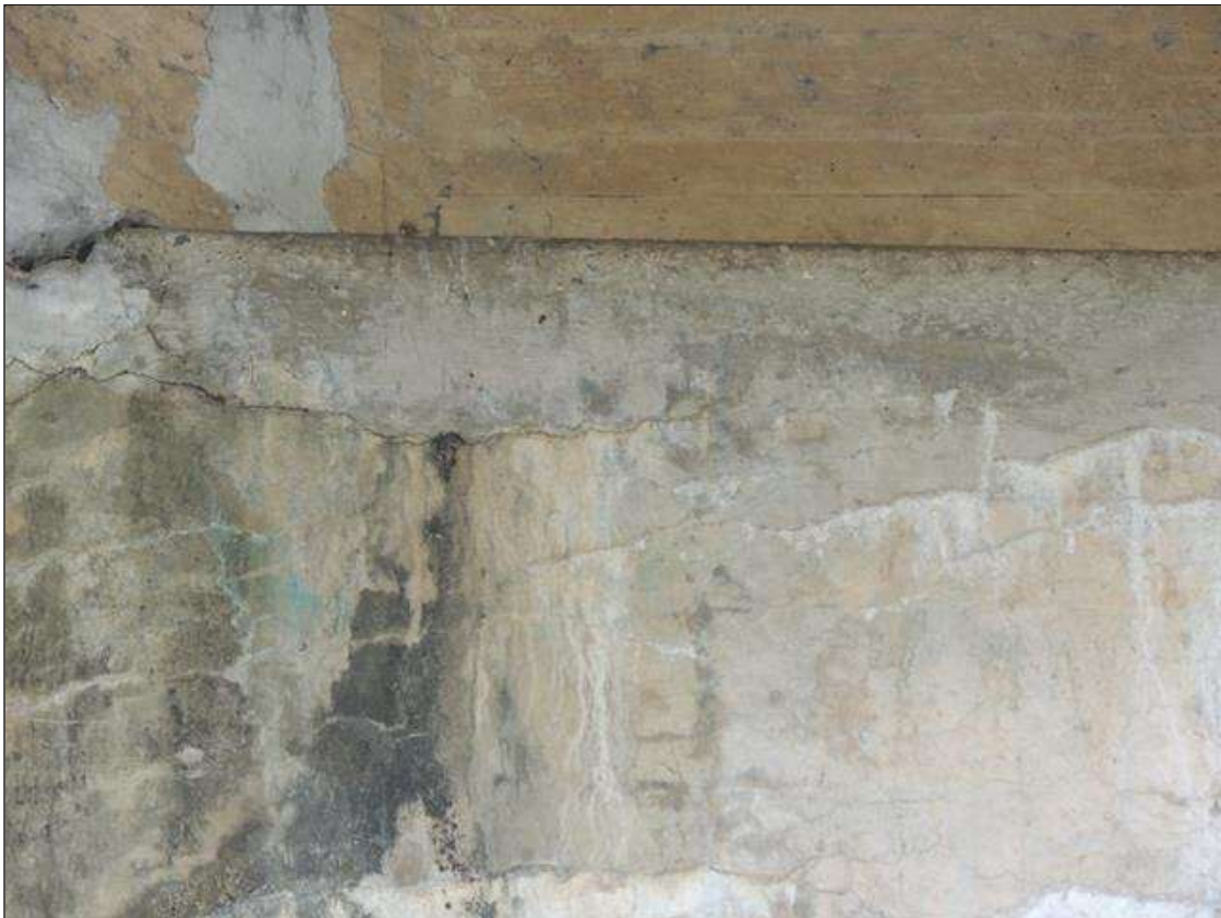
Bent 3 Cap : 4 Feet of Delamination/Spall/Patched Area: Delaminated. Spall 1 inch or less deep or 6 inches or less in diameter. SOUTH FACE OF CAP IS PATCHED AND DELAMINATED RIGHT OF G 3 12" DOWN FACE 4' LONG.
