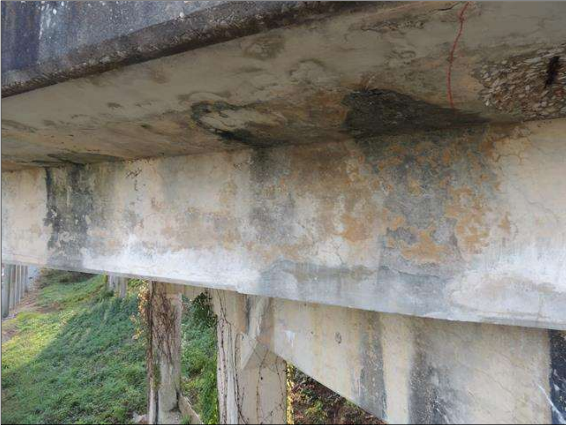
Span 4 Beam 4: 25 Feet of Cracking (RC and Other): Width 0.012-0.05 in. or spacing of 1.0-3.0 ft. RIGHT SIDE OF G 4 HAS SCATTERED MAP CRACKING IN FACE.
