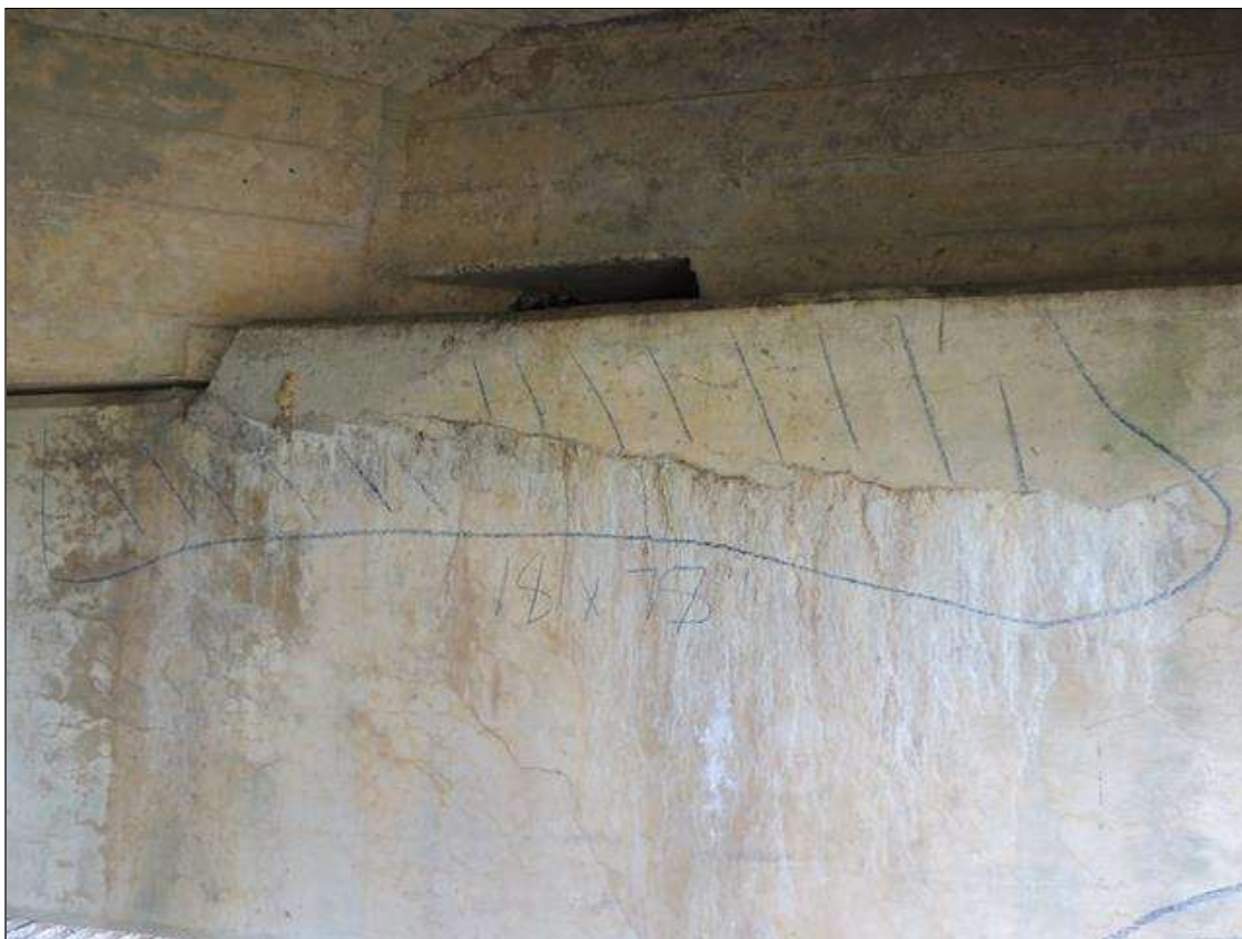
Bent 1 Cap : 7 Feet of Delamination/Spall/Patched Area: Delaminated. Spall 1 inch or less deep or 6 inches or less in diameter. Patched area that is sound BENT 1 SOUTH FACE OF CAP CRACKED PATCHED AND DELAMINATED AREA WITH HEAVY EFFLO FROM G2 OVER TO COL 2 18" DOWN FACE 78" LONG.
