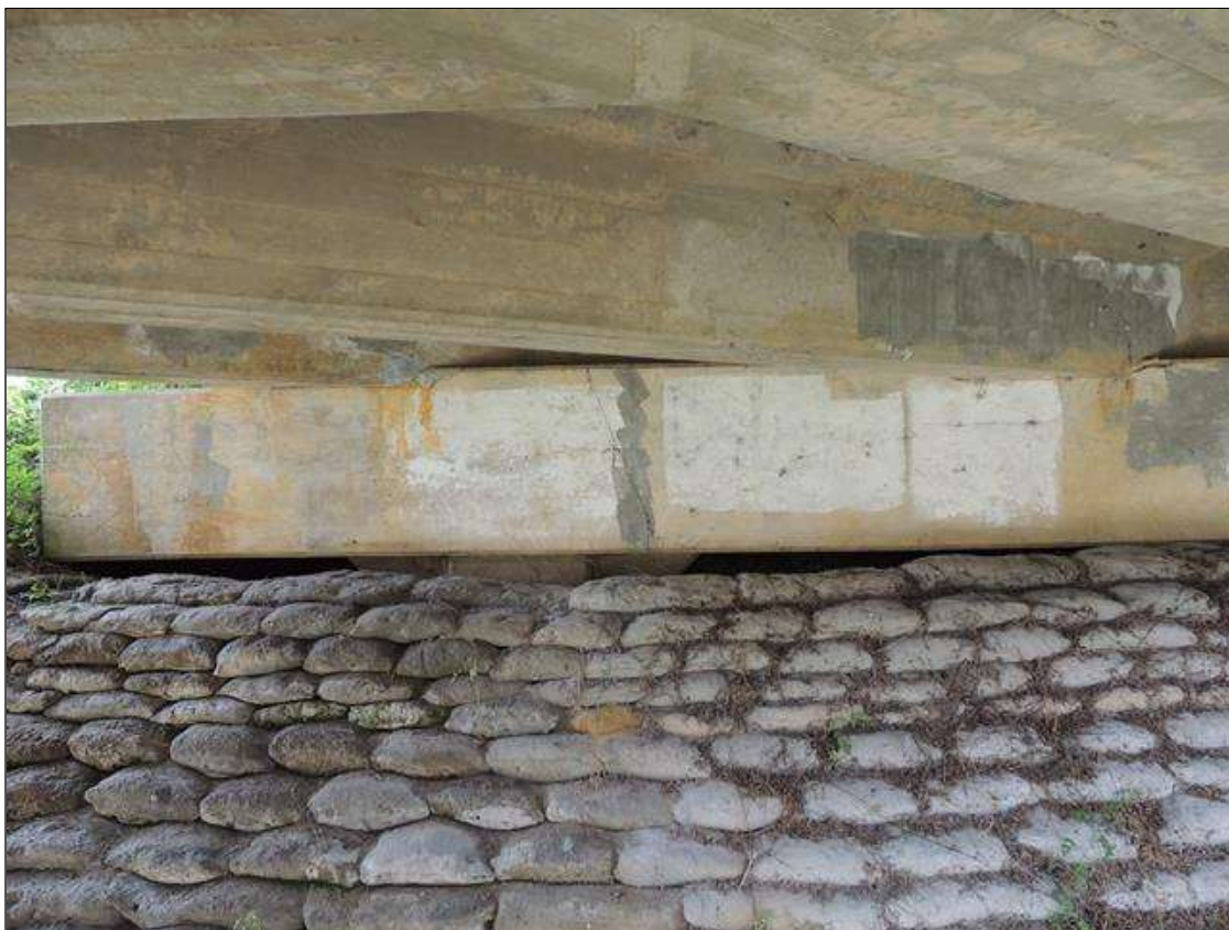
Bent 1 Cap : 45 Feet of Cracking (RC and Other): Width 0.012-0.05 in. or spacing of 1.0-3.0 ft. END BENT 1 HAS SCATTERED MAP CRACKING WITH HORIZ CRACKS FROM LEFT TO RIGHT END.
