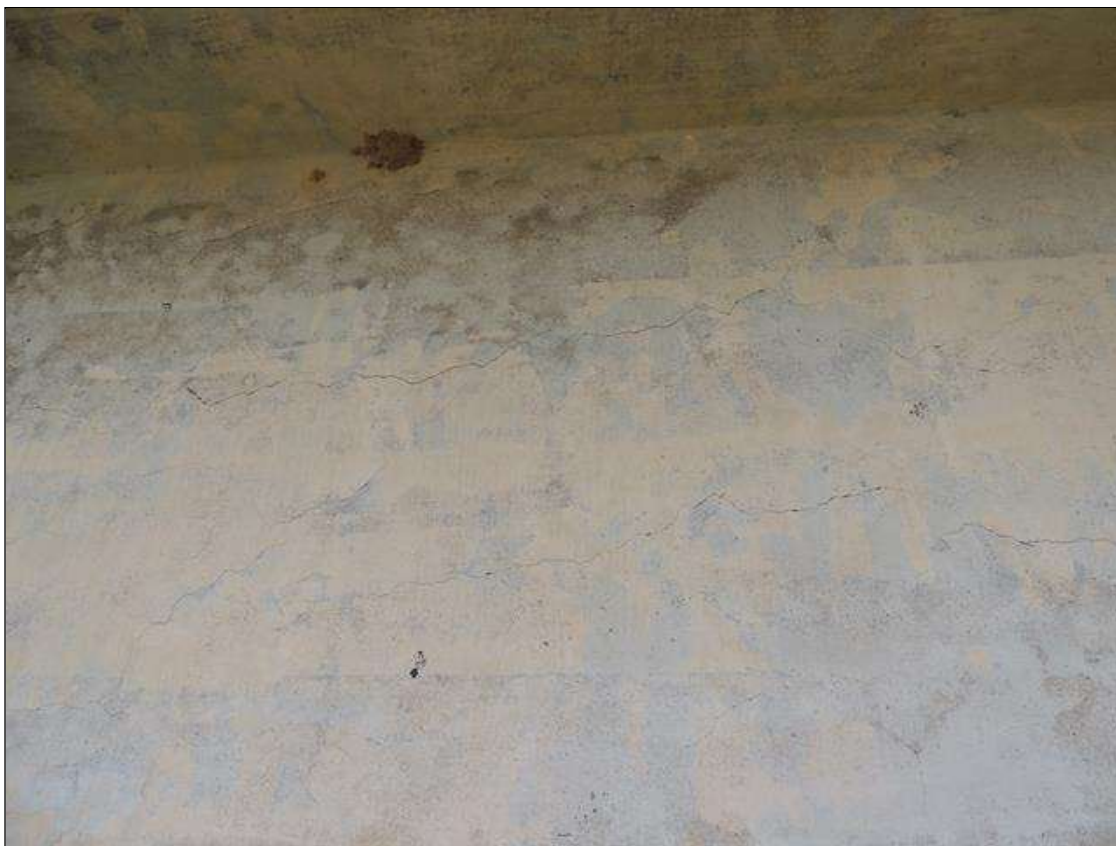
Span 1 Beam 1: 8 Feet of Cracking (RC and Other): Width 0.012-0.05 in. or spacing of 1.0-3.0 ft. SPAN 1 LEFT SIDE OF G1 NEAR BENT 1 SCATTERED MAP CRACKING IN FACE OF GIRDER.
