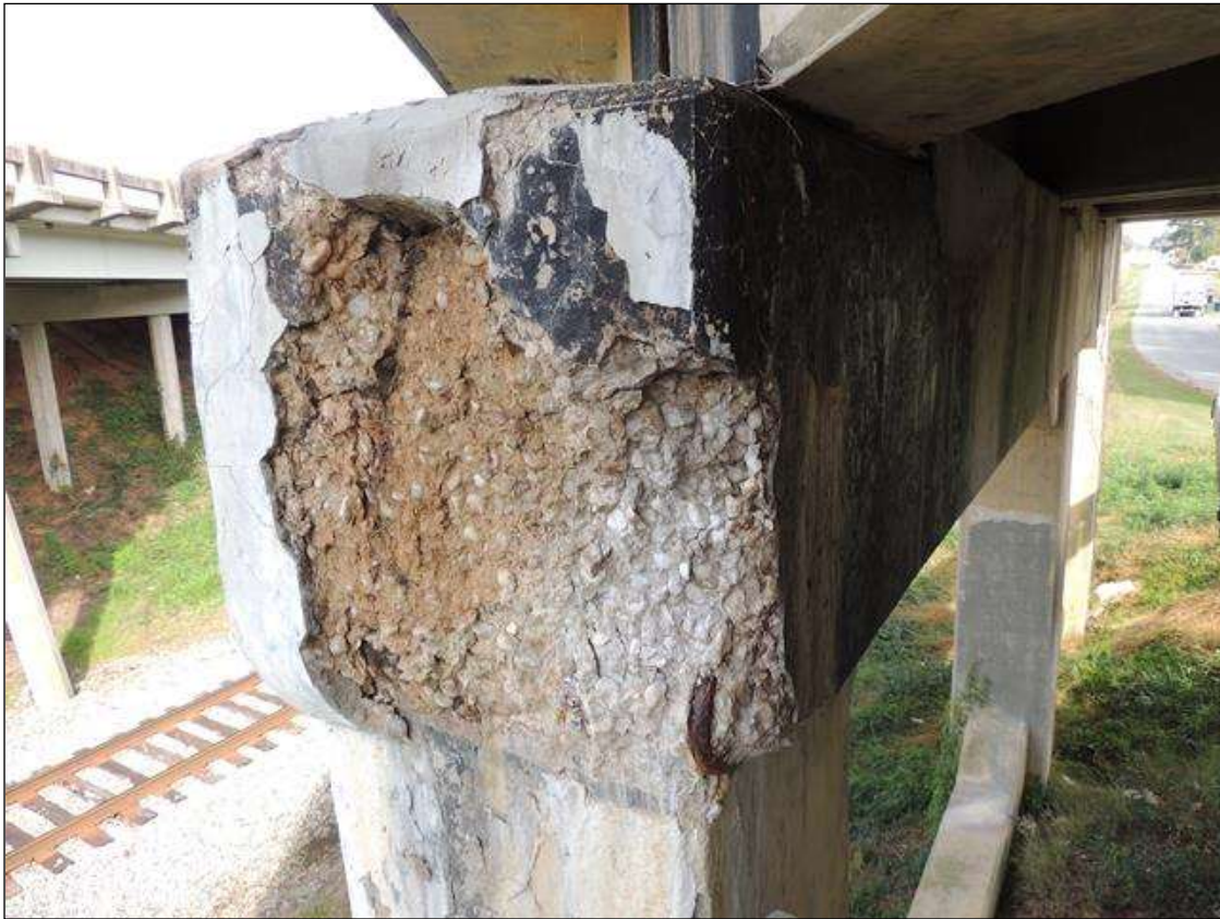
LEFT END OF BENT 1 CAP AND SOUTH FACE . SPALLED, CRACKED , DELAM. & DETERIORATED FROM LEFT END OUT 4' LONG X 38" WIDE X 3' TOP AND BOTTOM WITH REBAR.
