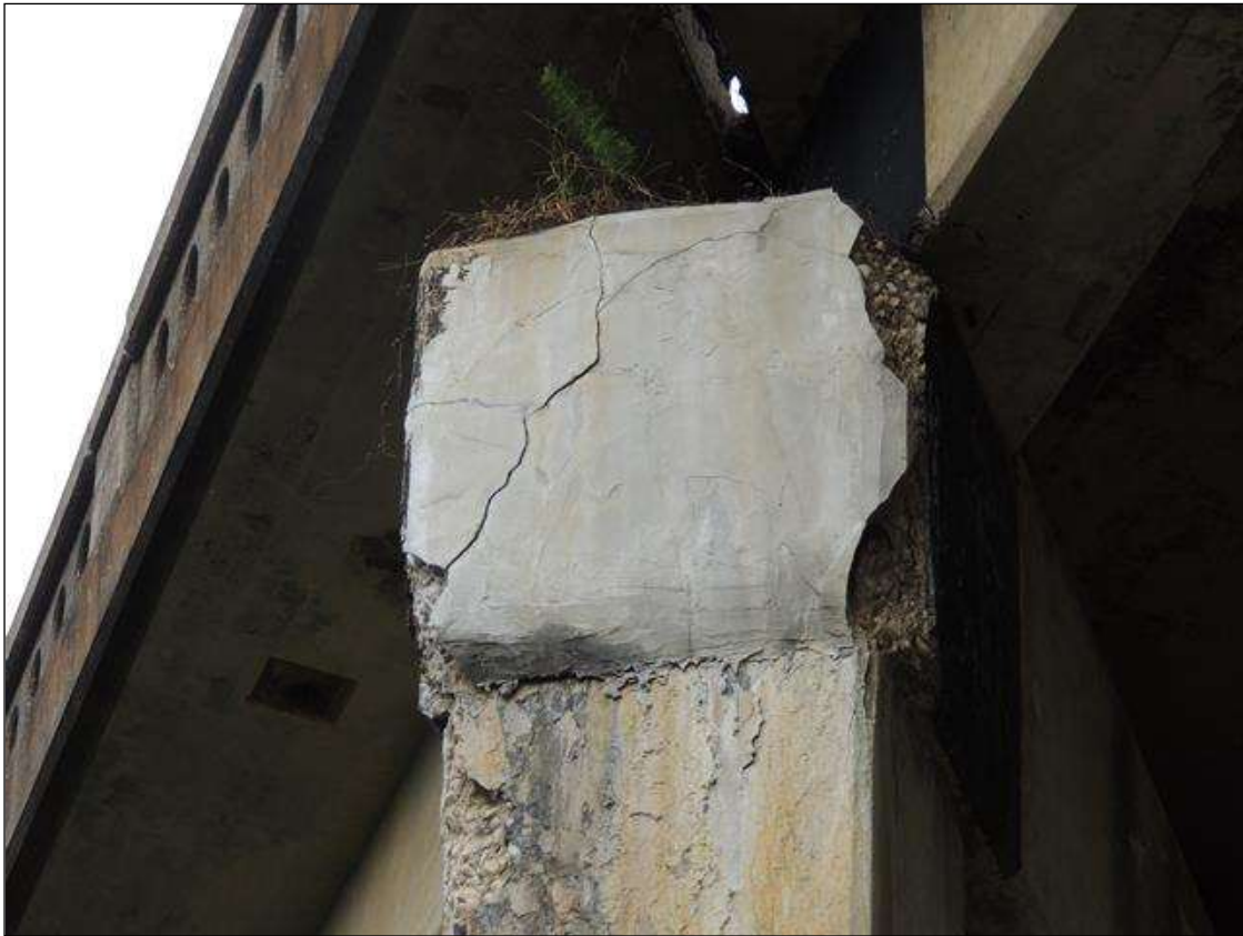
BT. 3 CAP LT. END CRACKED, SPALLED, DELAM.& DETERIORATED. 37" X 37" 3' ON N. & S. FACE 5" DEEP.
