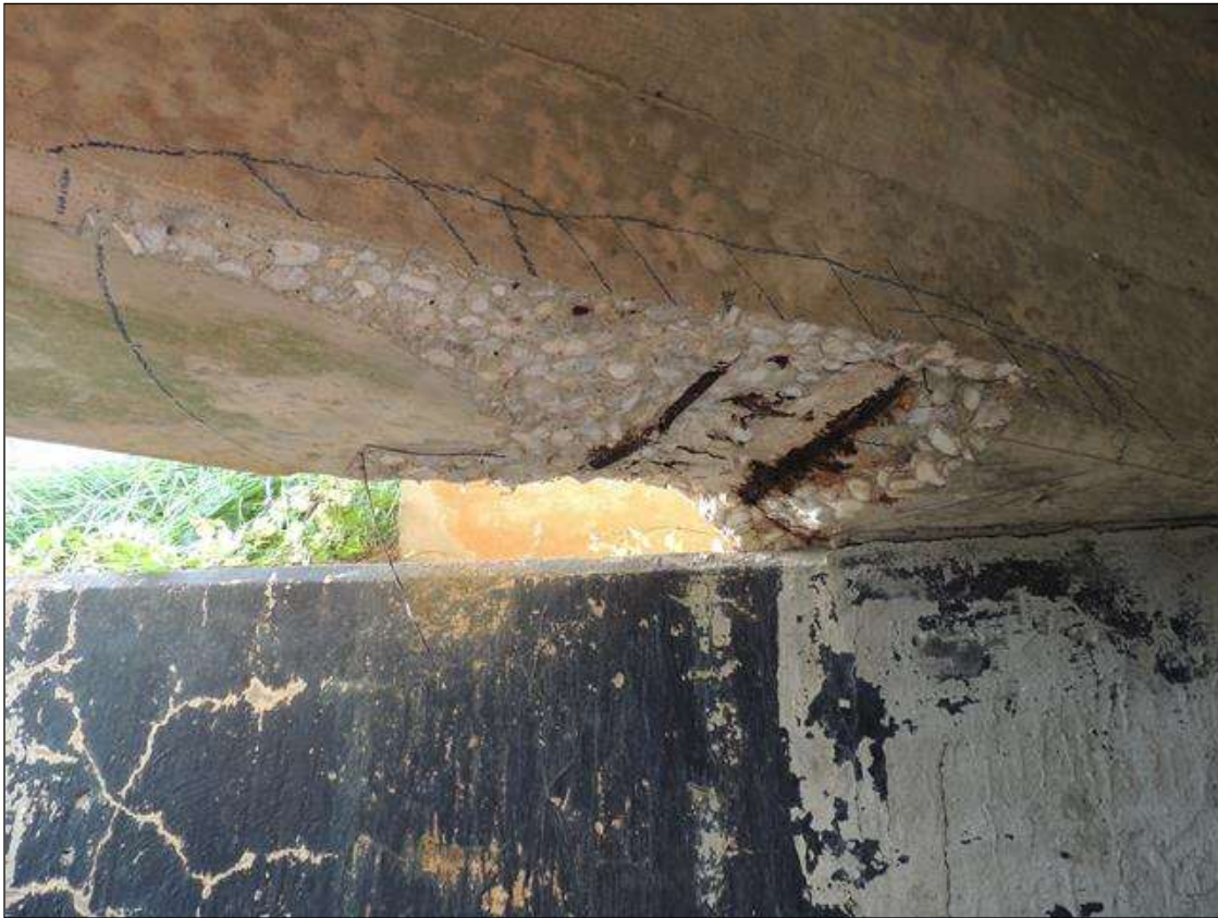
SPAN 5 G1 @ END BENT 2 SPALLED , DELAM. AND CRACKED 32" X 2 1/2" X 18"
