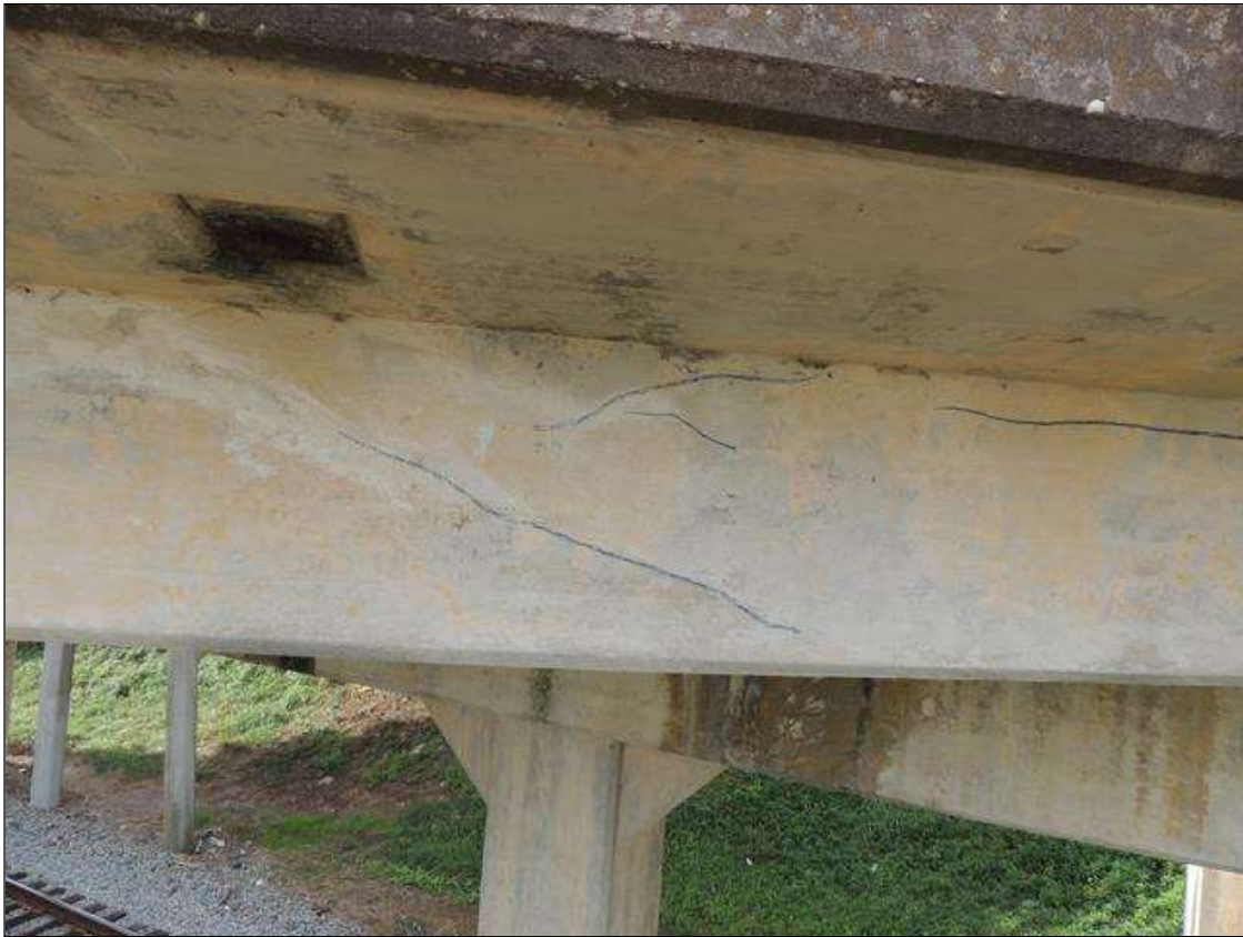
Span 2 Beam 4: 20 Feet of Cracking (RC and Other); Width 0.012-0.05 in. or spacing of 1.0-3.0 ft. SPAN 2 RIGHT SIDE OF G4 SCATTERED LONGITUDINAL CRACKS AND MAP CRACKING.
