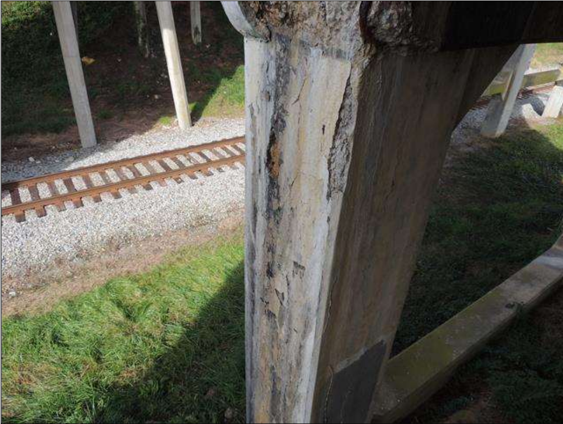
Bent 1 Pile 1: 1 Each of Delamination/Spall/Patched Area: Spall greater than 1 in. deep or greater than 6 in. diameter. Patched area that is unsound or showing distress. Does not warrant structural review. BENT 1 COL 1 WEST FACE END BENT 1 CRACKED SPALL DELAMINATED AND DETERIORATED 31" WIDE FROM TOP TO GROUND LINE 13' WITH HEAVY EFFLO EXPOSED. ALSO CRACKED AND DELAMINATED ON NORTH FACE AND SOUTH FACE 10".
