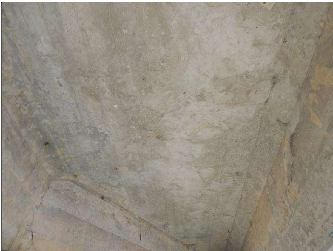
Span 4 Deck: 200 Square Feet of Delamination/Spall: Delaminated. Spall 1 in. or less deep or 6 in. or less in diameter. BOTTOM OF DECK IN BAY 3 HAS A SMALL PATCHED AREA WITH SOME DELAMINATION. BAYS 1 & 2 HAVE SIMILAR AREAS.
