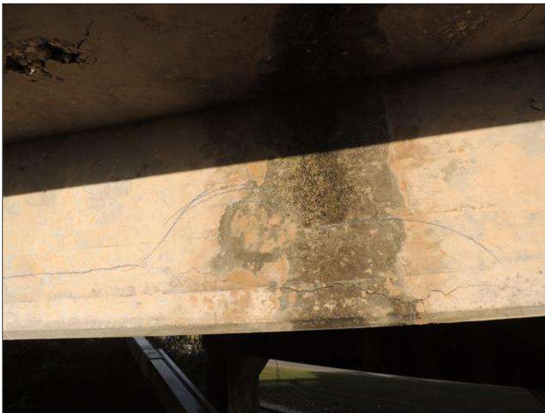
Span 5 Beam 1: 10 Feet of Cracking (RC and Other): Width 0.012-0.05 in. or spacing of 1.0-3.0 ft. G1 LEFT FACE NEAR MID SPAN IS CRACKED.
