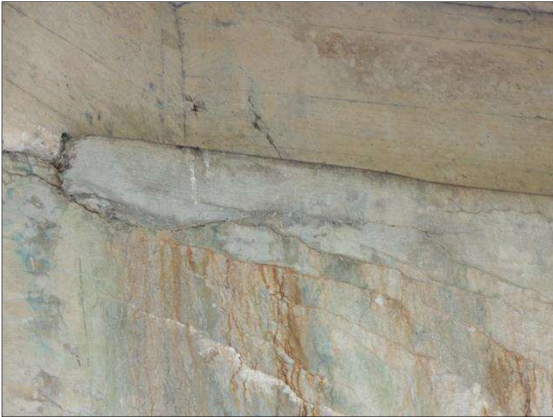
Bent 3 Cap : 3 Feet of Delamination/Spall/Patched Area: Delaminated. Spall 1 inch or less deep or 6 inches or less in diameter. SOUTH FACE OF CAP IS PATCHED AND DELAMINATED RIGHT OF G 2 10" DOWN FACE 36" LONG.
