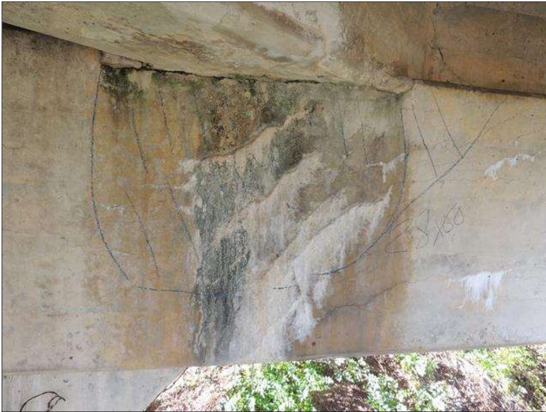
Bent 4 Cap : 5 Feet of Delamination/Spall/Patched Area: Delaminated. Spall 1 inch or less deep or 6 inches or less in diameter. SOUTH FACE OF CAP IS CRACKED AND DELAMINATED 28" UNDER G 3 AND DOWN FACE 5'.
