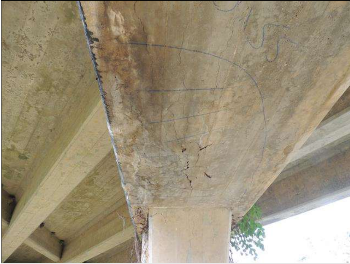
Bent 4 Cap : 15 Feet of Cracking (RC and Other): Width 0.012-0.05 in. or spacing of 1.0-3.0 ft. BOTTOM OF CAP BETWEEN COL. 1 7 COL. 2 CRACKED AND DELAMINATED WITH EFFLO 35" X 55".
