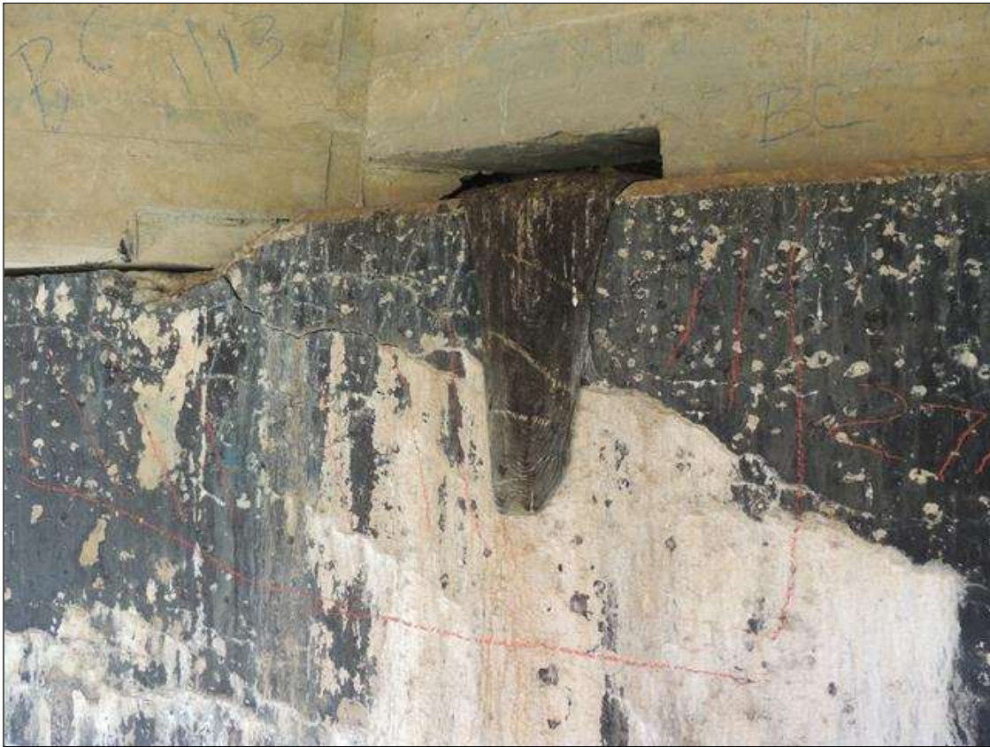
Bent 3 Cap : 5 Feet of Delamination/Spall/Patched Area: Delaminated. Spall 1 inch or less deep or 6 inches or less in diameter. NORTH FACE OF CAP IS CRACKED, SPALLED AND DELAMINATED WITH HEAVY EFFLO AT G 3. AREA IS 27" X 54"
