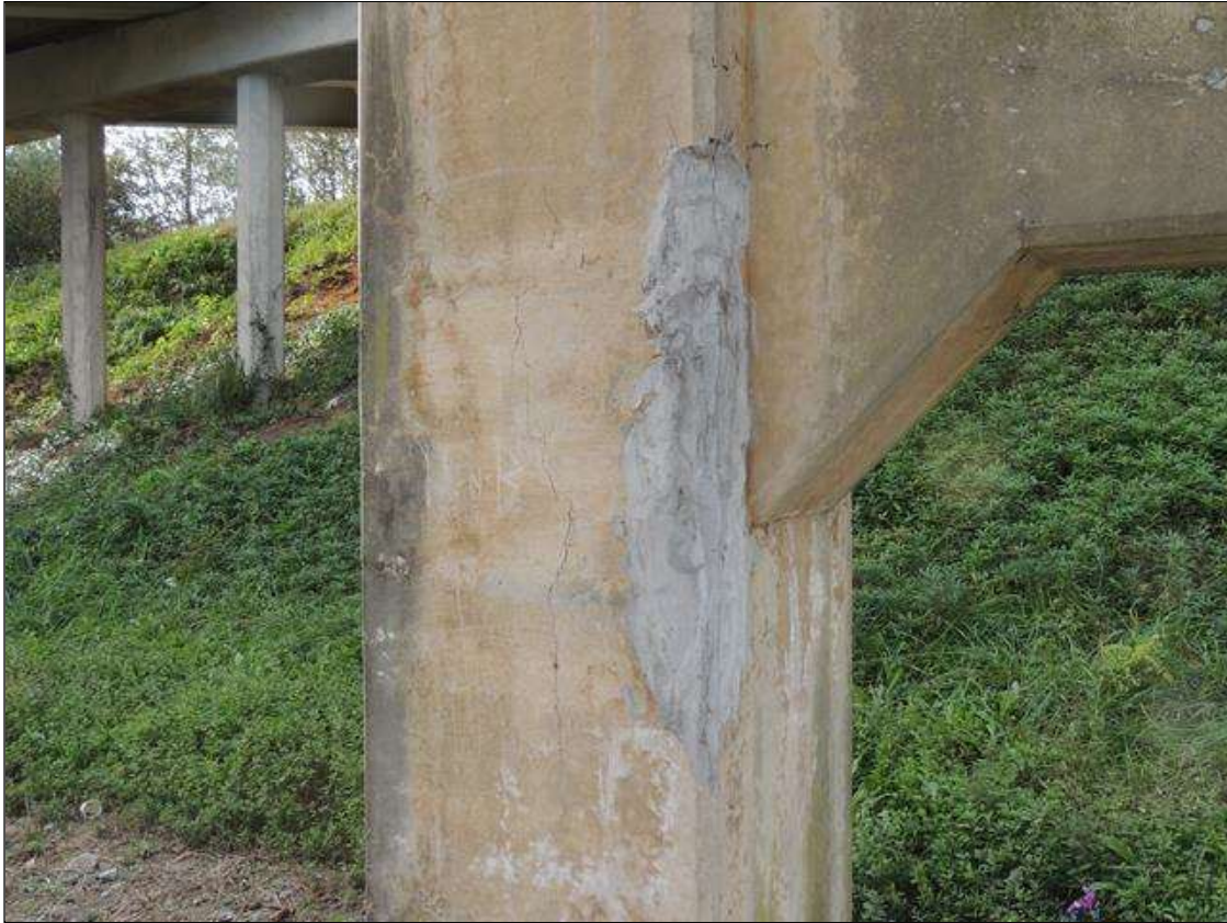
Bent 3 Pile 1: 0 Each of Delamination/Spall/Patched Area: Delaminated. Spall 1 in. or less deep or 6 in. or less in diameter. COL. 1 HAS A PATCHED AREA SOUTH EAST CORNER @ STRUT AREA IS 3' HIGH AND 4" ON EACH FACE.
