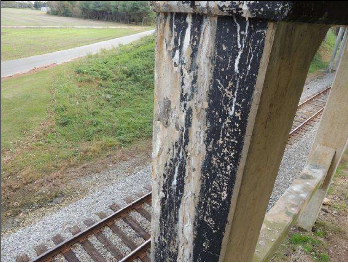
Bent 4 Pile 3: 1 Each of Delamination/Spall/Patched Area: Delaminated. Spall 1 in. or less deep or 6 in. or less in diameter. EAST FACE IS CRACKED FROM TOP DOWN 16' X 25" WIDE.
