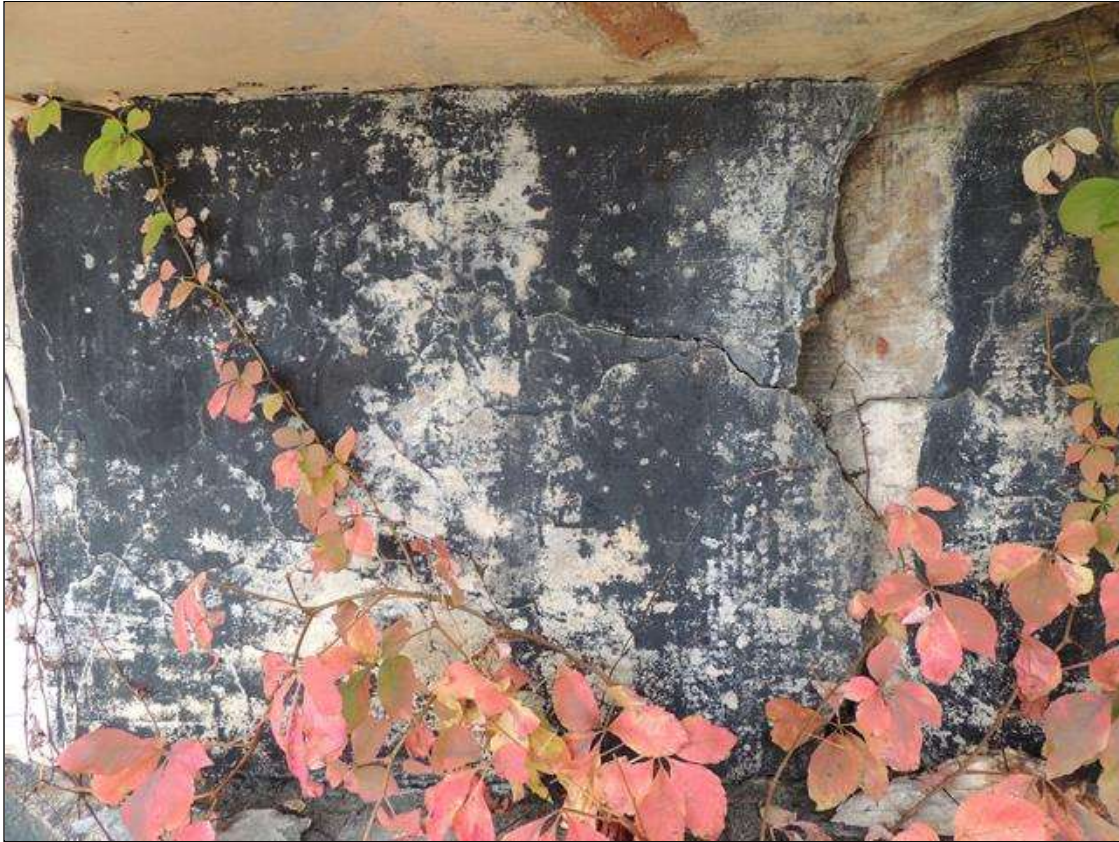
Span 1 Beam 4: 2 Feet of Delamination/Spall/Patched Area: Delaminated. Spall 1 in. or less deep or 6 in. or less in diameter. Patched area that is sound. SPAN 1 RIGHT SIDE OF G4 CRACKED SPALL DELAMINATED AREA FROM THE END BACK 20" TOP DOWN 24" 3" DEEP.
