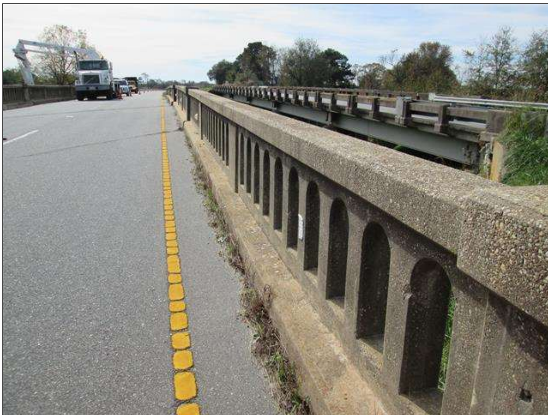
RAIL AND CURB LEFT SIDE SPAN 2. ( SIM IN ALL SPANS BOTH SIDES )
