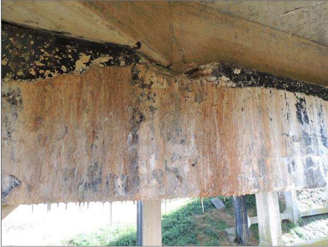
Bent 3 Cap : 10 Feet of Delamination/Spall/Patched Area: Spall greater than 1 inch deep or greater than 6 inches in diameter. NORTH FACE OF CAP IS CRACKED , SPALLED AND DELAMINATED WITH EXCESSIVE EFFLO FROM G 1 TO G 2 42" TOP TO BOTTOM 10' LONG. SPALLED AREA IS 11" X 27" X 9" DEEP.
