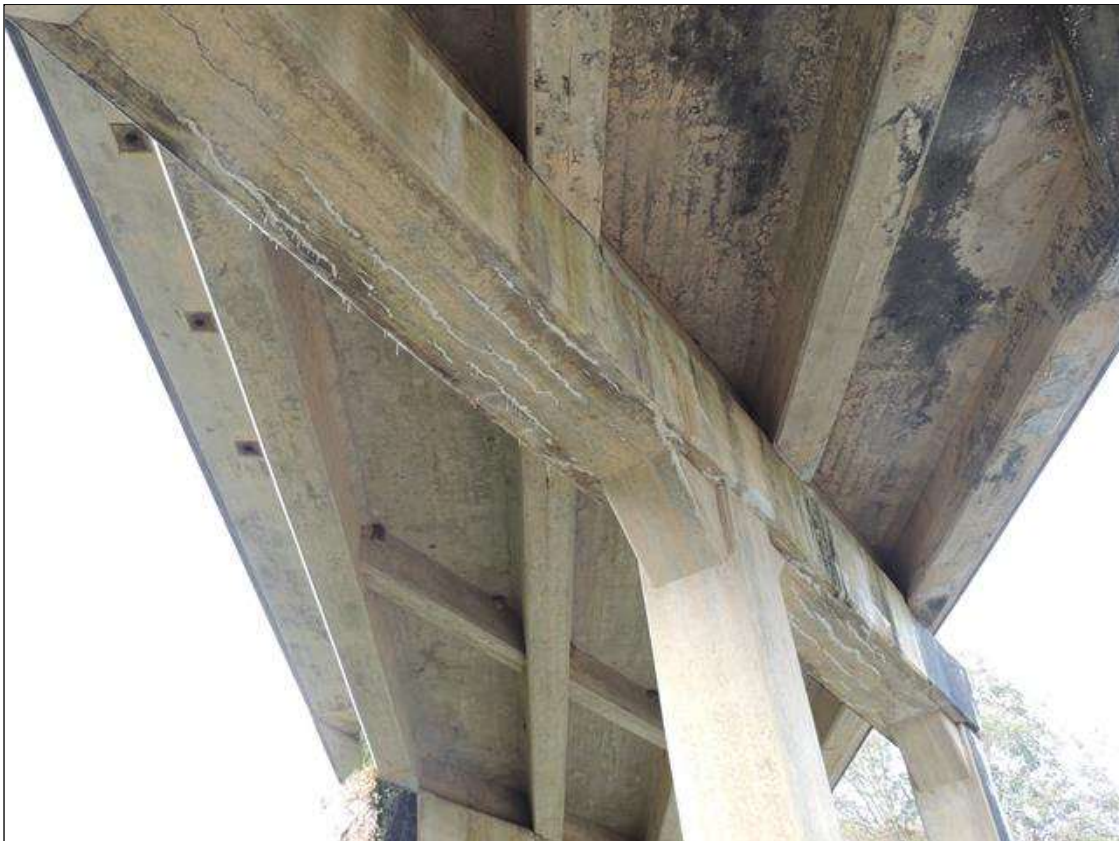
Bent 3 Cap : 0 Feet of Cracking (RC and Other): Width greater than 0.05 in. or spacing of less than 1 ft. BOTTOM OF CAP BETWEEN COL. 1 & 2 AND COL. 3 & 4 HAVE AREAS OF HEAVY MAP CRACKING WITH EFFLO.
