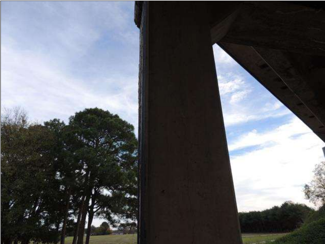
Bent 4 Pile 3: 0 Each of Cracking (RC and Other): Width 0.012-0.05 in. or spacing or 1.0-3.0 ft. NORTH FACE HAS SCATTERED VERTICAL AND MAP CRACKING WITH SOME DELAMINATION. SIMILAR IN OTHER FACES.
