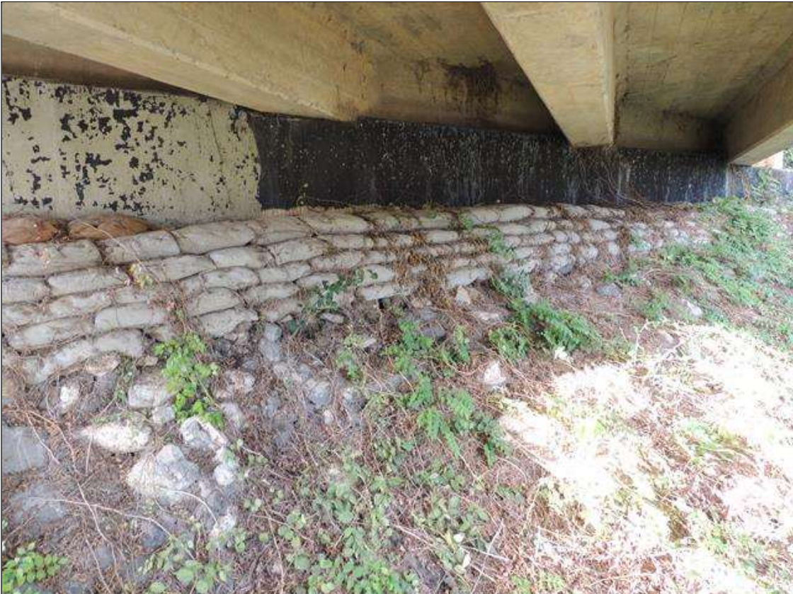
End Bent 2 Cap : 45 Feet of Cracking (RC and Other): Width 0.012-0.05 in. or spacing of 1.0-3.0 ft. FACE OF END BENT 2 CAP HAS SCATTERED MAP CRACKING FROM LEFT END TO RIGHT END.
