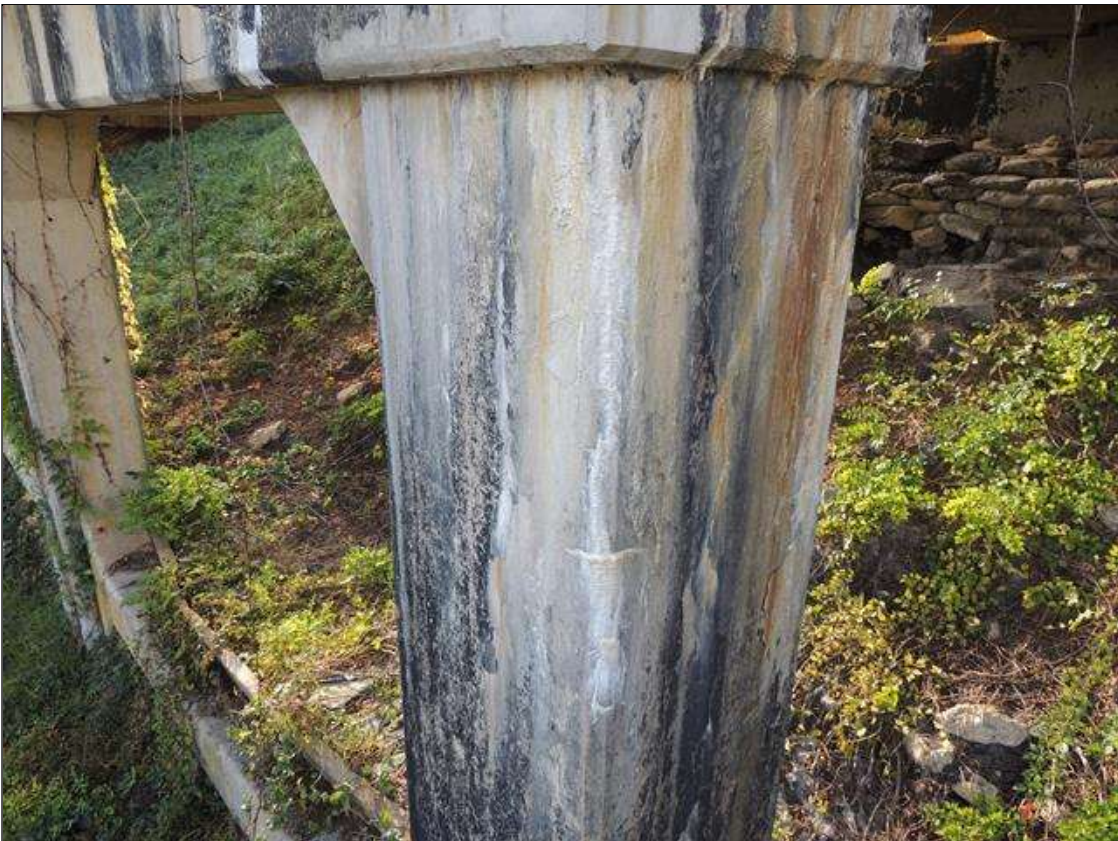
Bent 4 Pile 3: 0 Each of Cracking (RC and Other): Width 0.012-0.05 in. or spacing or 1.0-3.0 ft. SOUTH AND EAST FACES OF COL. 3 HAVE CRACKS WITH HEAVY EFFLO FROM CAP DOWN 10'. OTHER FACES ARE CRACKED.
