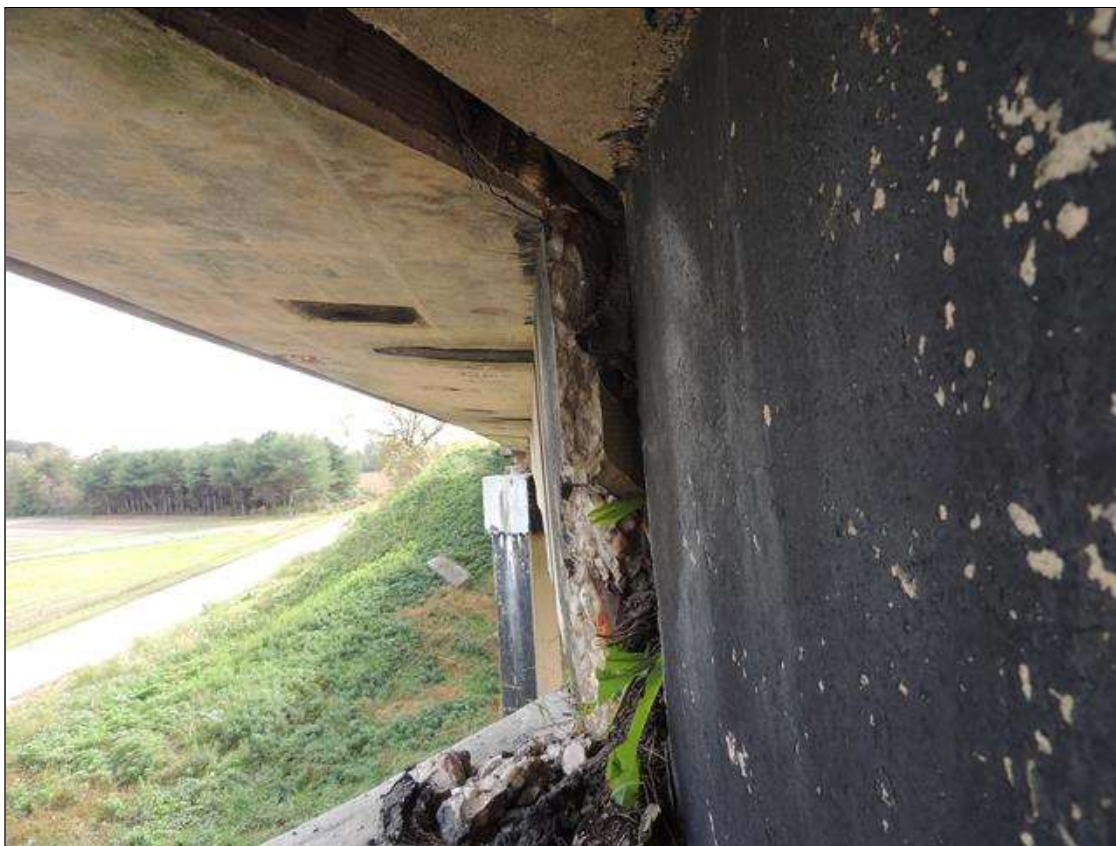
SPAN 3 HAS SHIFTED 3" TO EAST OVER BENT 3.
