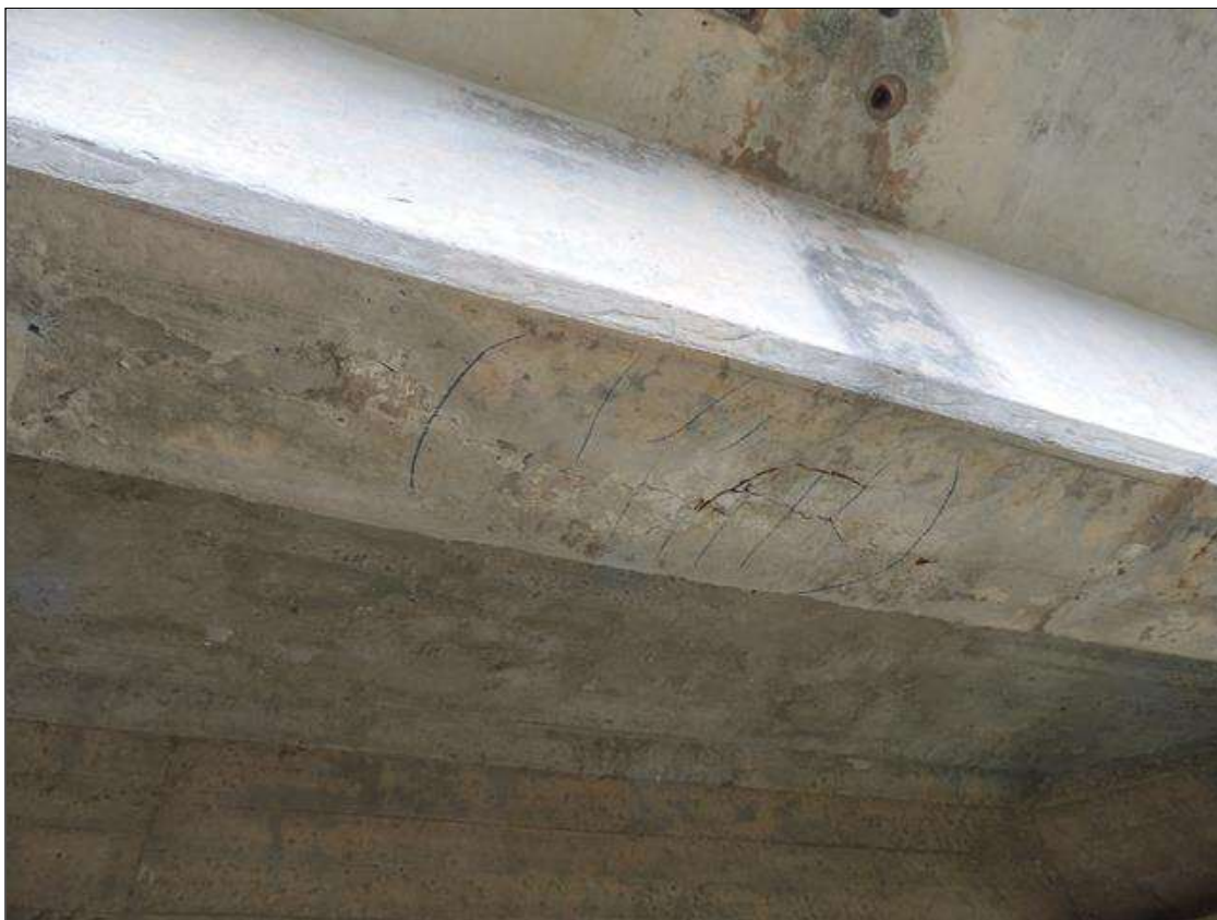
Span 2 Beam 1: 3 Feet of Delamination/Spall/Patched Area: Delaminated. Spall 1 in. or less deep or 6 in. or less in diameter. Patched area that is sound. SPAN 2 G1 CRACKED AND DELAMINATED AREA NEAR MID SPAN 18" UNDER BOTTOM 5" UP RIGHT FACE 32" LONG.
