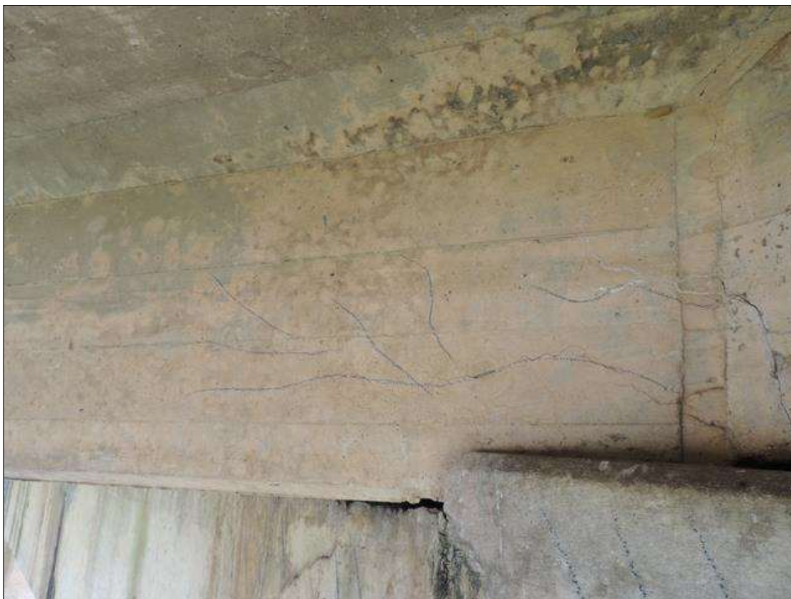
Span 2 Beam 3: 5 Feet of Cracking (RC and Other): Width 0.012-0.05 in. or spacing of 1.0-3.0 ft. SPAN 2 RIGHT SIDE OF G3 SCATTERED MAP CRACKING AT BENT 2.
