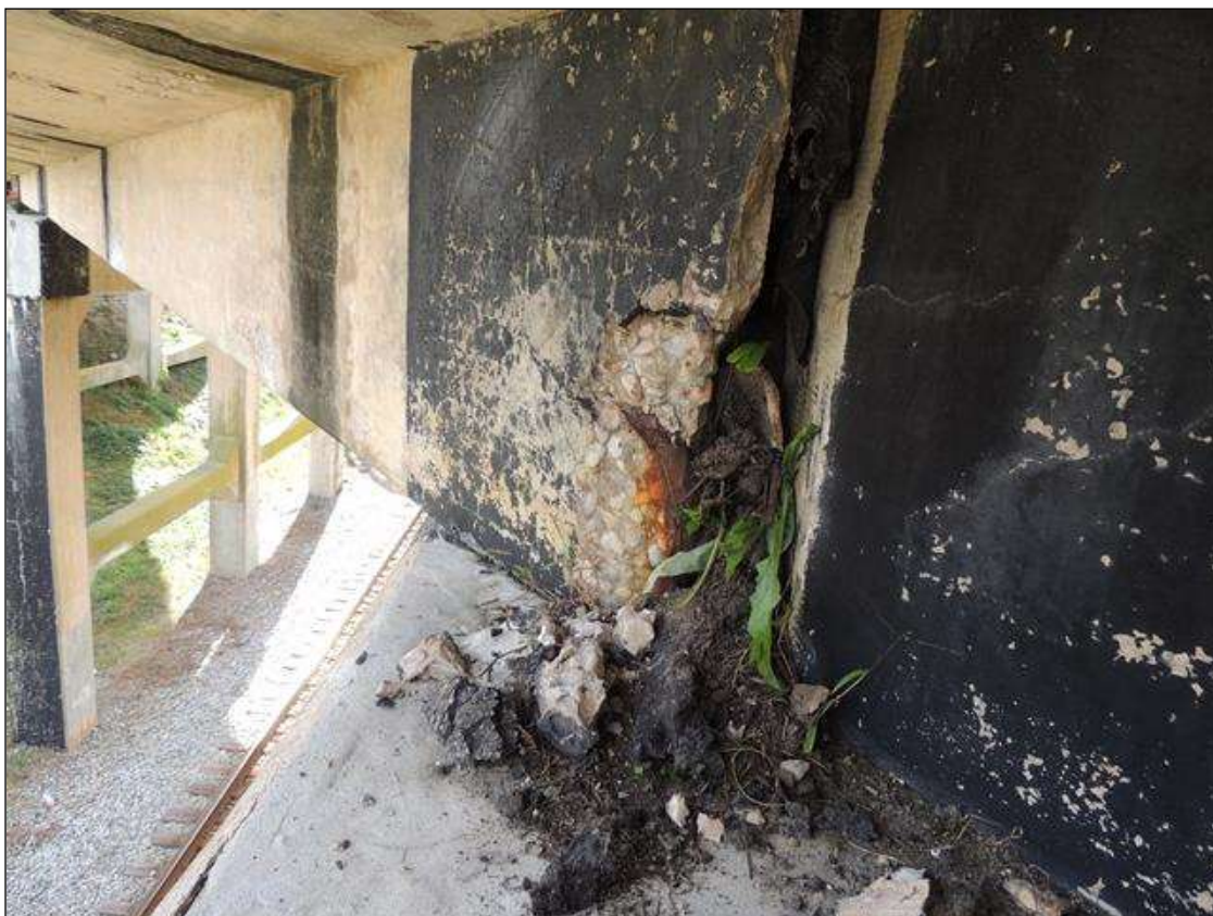
SP. 3 RT. SIDE G 4 DELAM. & SPALLED AREA OVER BT. 3 9" X 24" WITH LARGE REBAR EXPOSED.
