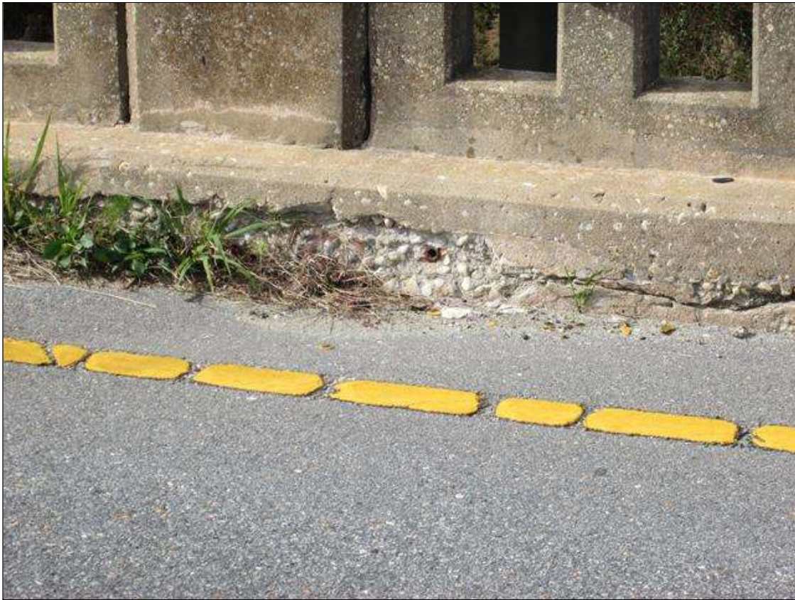
Span 1 Left Bridge Rail: 4 Feet of Delamination/Spall/Patched Area: Delaminated. Spall 1 in. or less deep or 6 in. or less in diameter. Patched area that is sound. LEFT CURB @ MID SPAN FACE IS CRACKED , SPALLED AND DELAMINATED. AREA IS 4' LONG 6" HIGH 1" DEEP.
