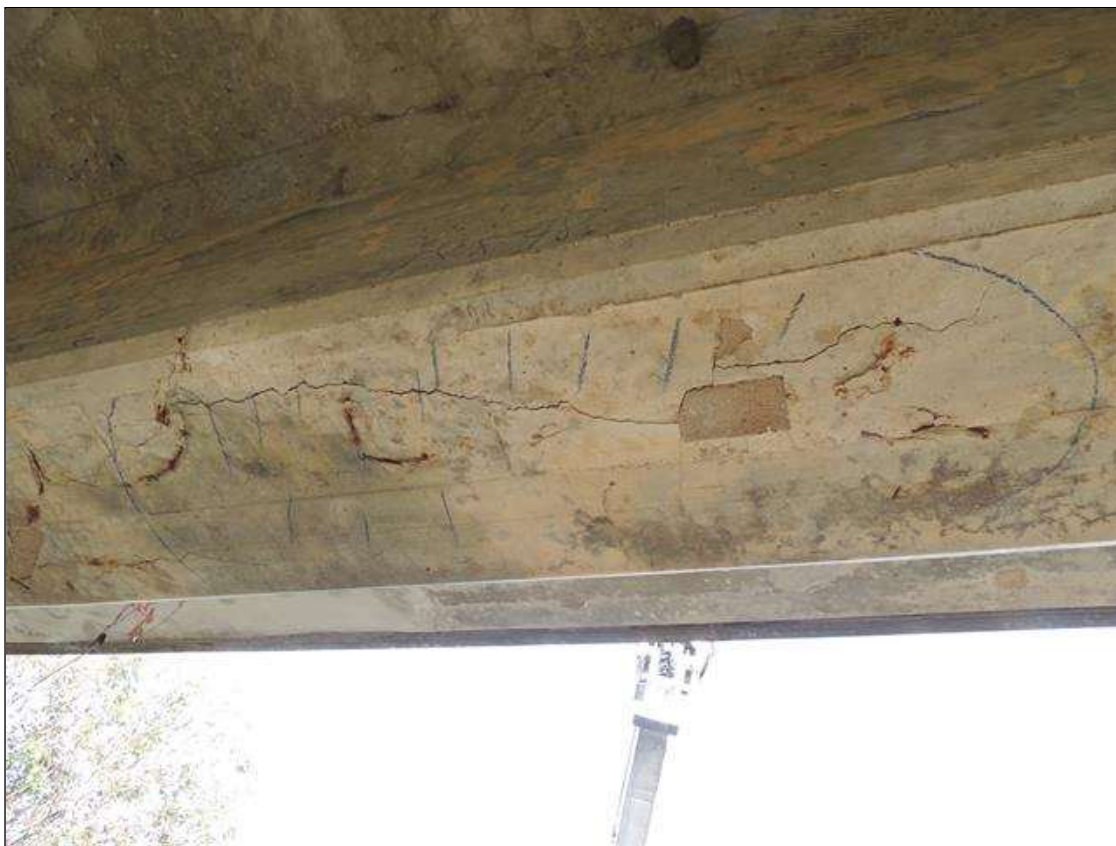
Span 4 Beam 4: 4 Feet of Delamination/Spall/Patched Area: Delaminated. Spall 1 in. or less deep or 6 in. or less in diameter. BOTTOM OF G 4 IS CRACKED & DELAMINATED 7' FROM BENT 4 18" UNDER BOTTOM 4' LONG.
