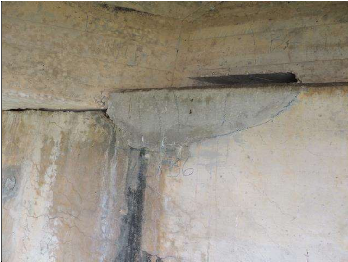
Bent 2 Cap : 3 Feet of Delamination/Spall/Patched Area: Delaminated. Spall 1 inch or less deep or 6 inches or less in diameter. Patched area that is sound BENT 2 SOUTH FACE OF CAP CRACKED AND DELAMINATED AND PATCHED AREA RIGHT SIDE OF G2 12" X 36".
