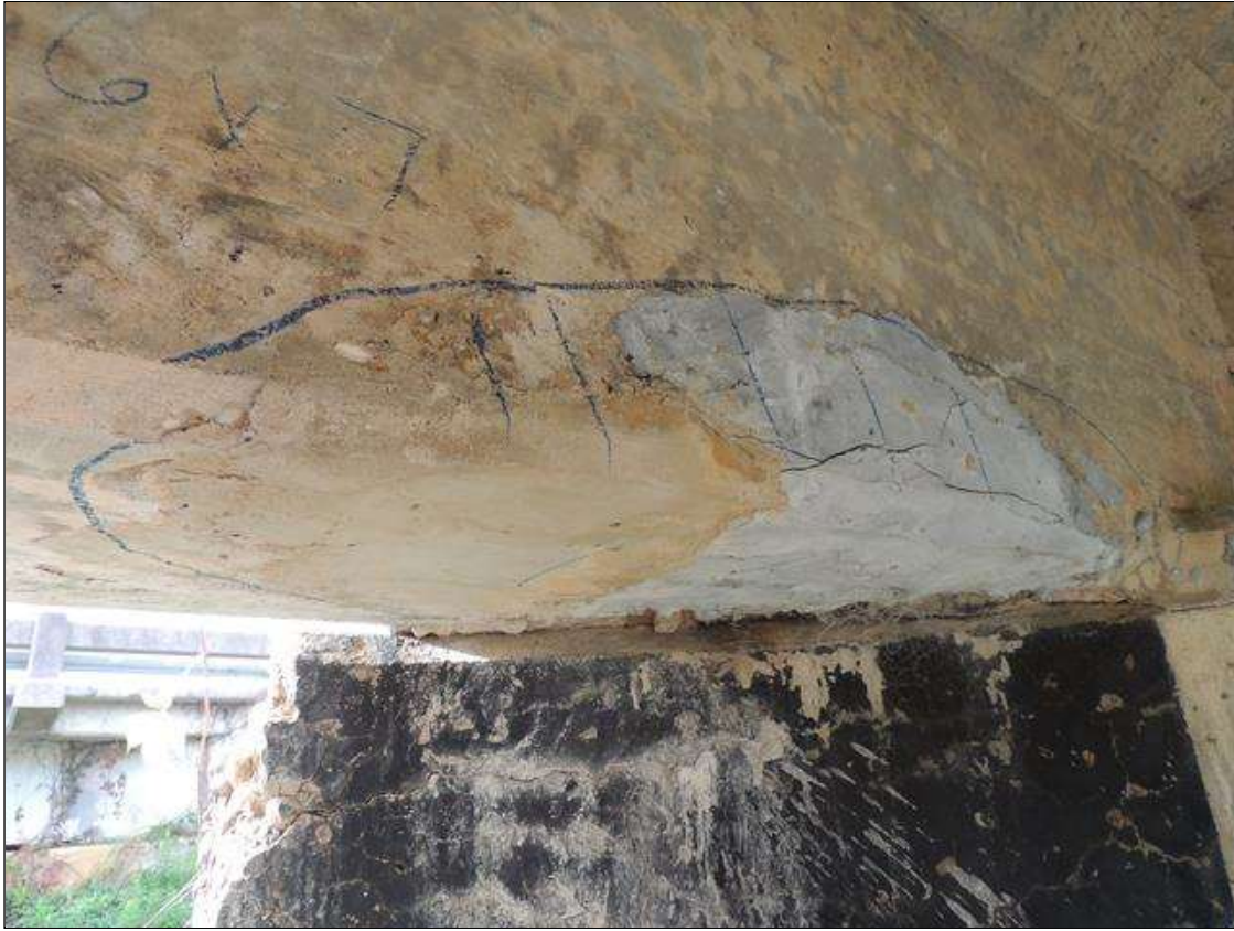
Span 4 Beam 1: 3 Feet of Delamination/Spall/Patched Area: Delaminated. Spall 1 in. or less deep or 6 in. or less in diameter. RIGHT SIDE AND BOTTOM OF G1 AT BENT 4 PATCHED AREA IS DELAMINATED 16" UNDER BOTTOM 3' LONG & 7" UP FACE.
