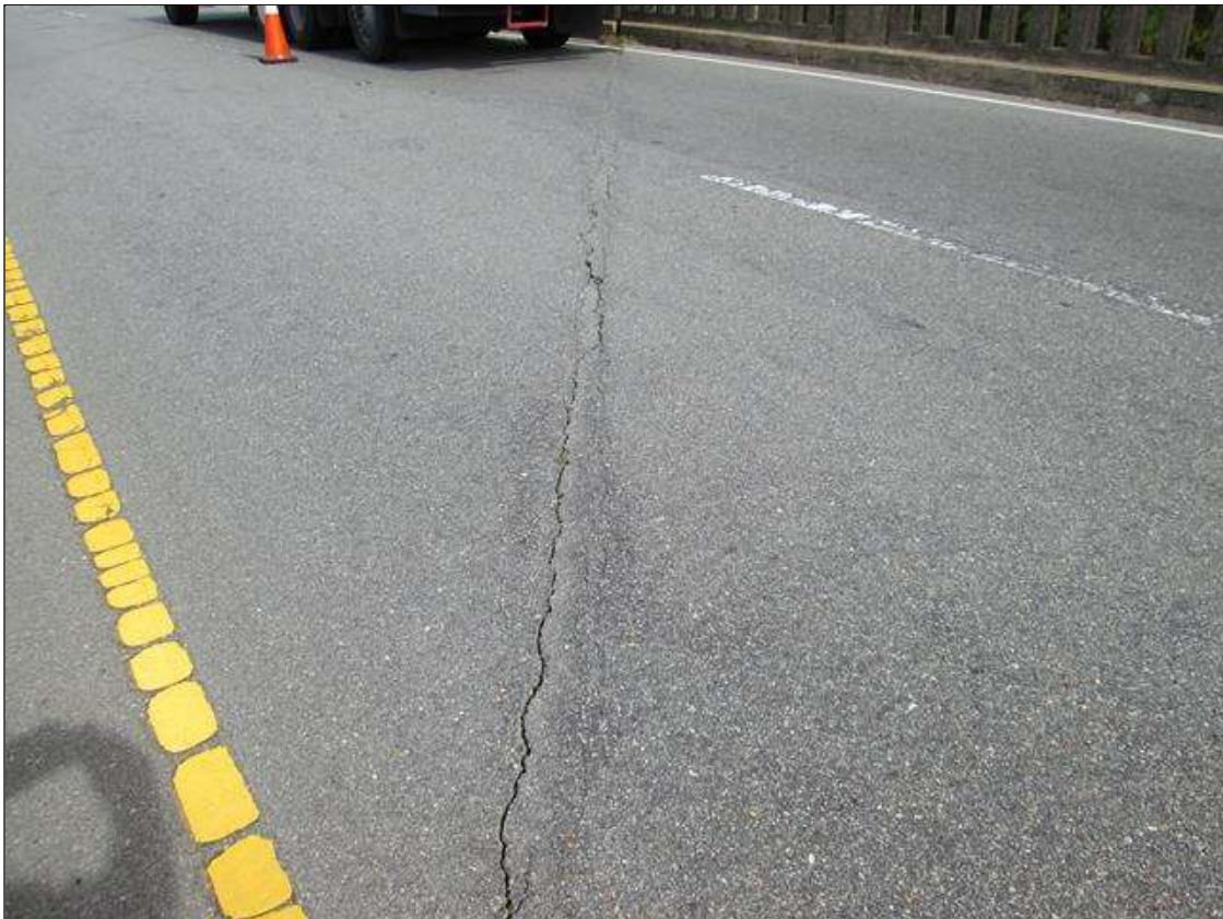
Expansion Joint 2 : 42 Feet of Seal Cracking: Surface crack. ASPHALT OVER BENT 1 JOINT IS CRACKED.
