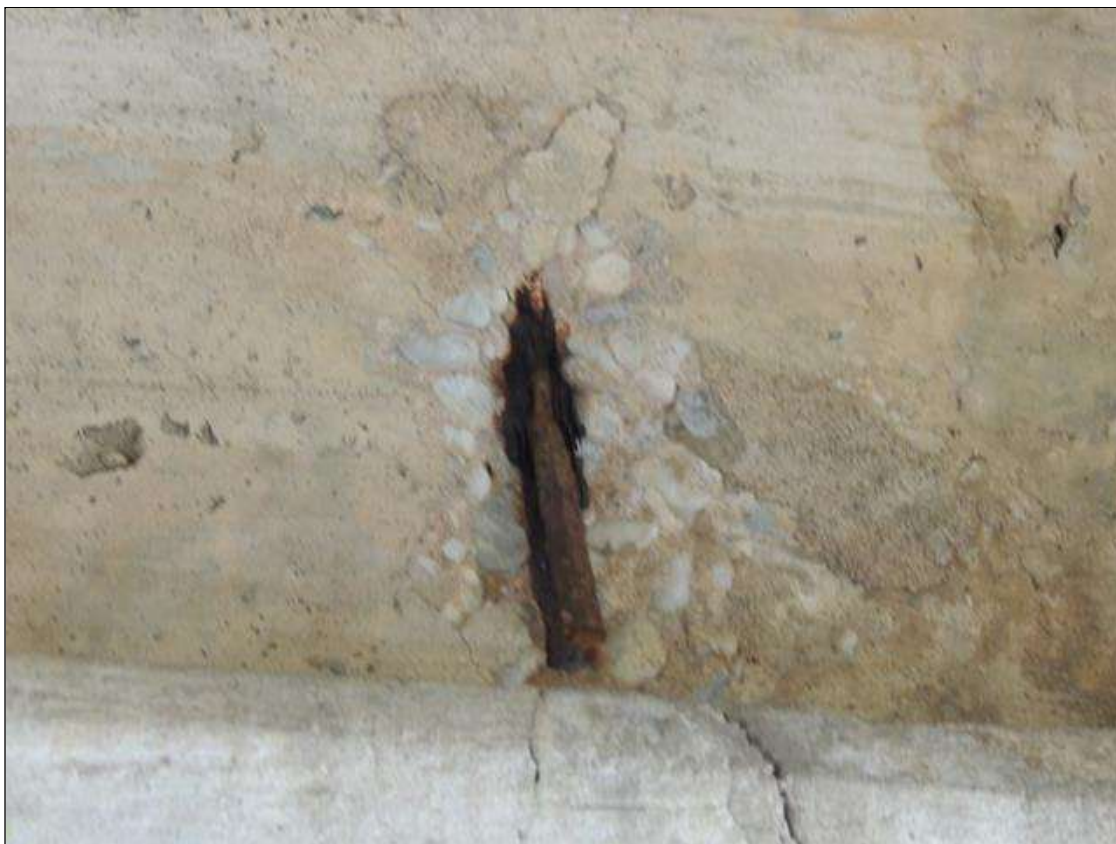
END DIAPHRAGM OVER BENT 1 IN BAY 1 6" X 8" X 3/4" VERTICAL REBAR EXPOSED.
