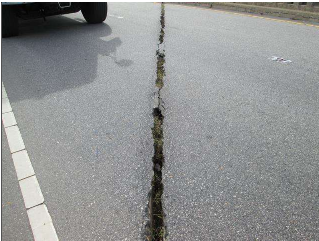
Expansion Joint 4 : 35 Feet of Leakage: Moderate. More than a drip and less than free flow of water. 35' OF JOINT MATERIAL AND ASPHALT MISSING OVER BENT 3.
