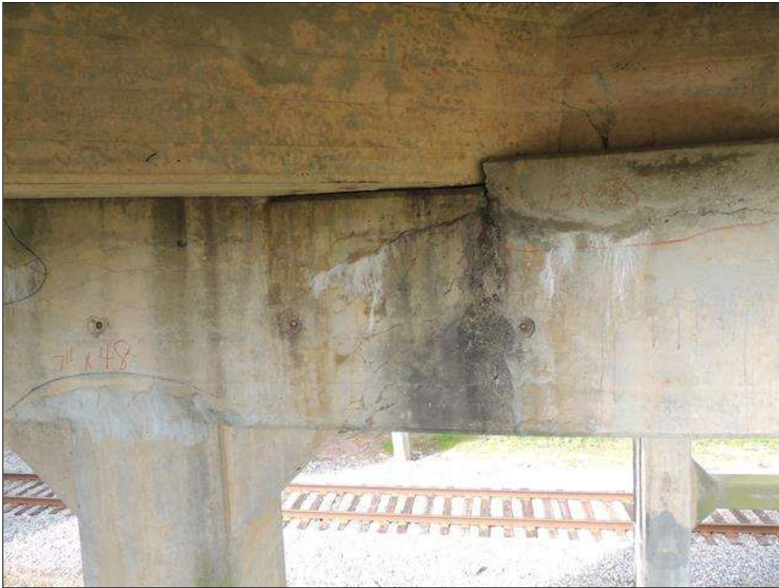
Bent 1 Cap : 0 Feet of Cracking (RC and Other): Width greater than 0.05 in. or spacing of less than 1 ft. BENT 1 SOUTH FACE OF CAP HAS SCATTERED MAP CRACKING AND HORIZ CRACKS FROM LEFT TO RIGHT END WITH EFFLO STAINS LEACHING.
