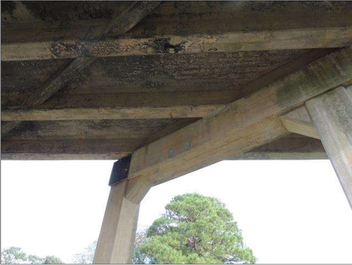
Bent 2 Cap : 0 Feet of Delamination/Spall/Patched Area: Delaminated. Spall 1 inch or less deep or 6 inches or less in diameter. NORTH FACE OF CAP HAS 3 PATCHED AREAS IN FACE AT G 3.
