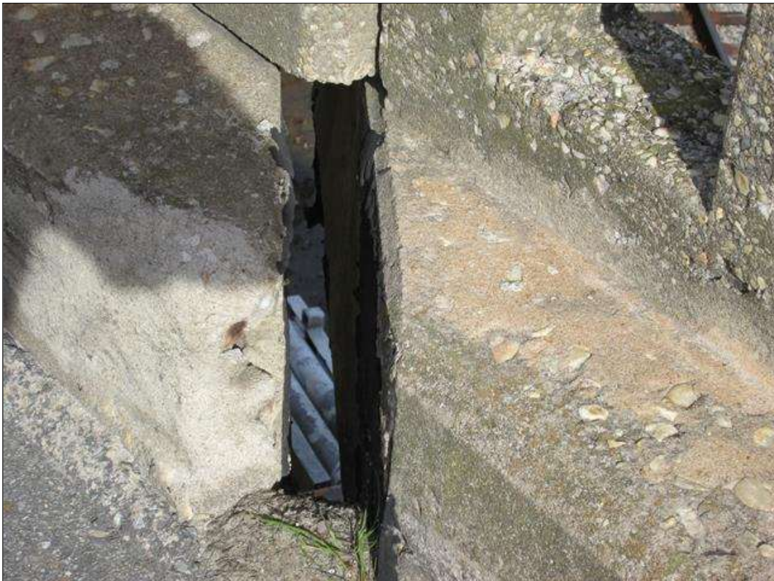
Expansion Joint 4 : 0 Feet of Leakage: Free flow of water through the joint. JOINT MATERIAL MISSING IN RIGHT CURB AREA OVER BENT 3. OPENING IS 2 1/2" WIDE SPANS ARE MISSALINGED
