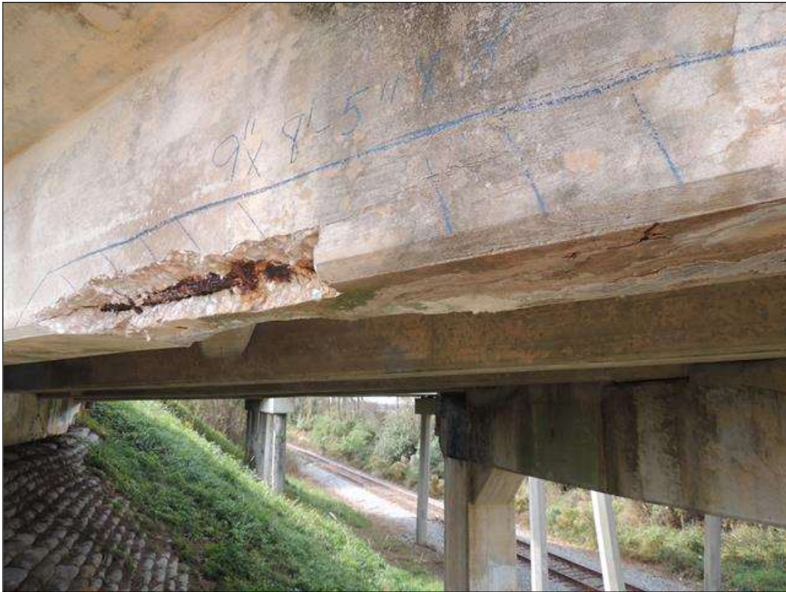
SPAN 1 G4 CRACKED SPALLED AND DELAMINATED AREA ALONG BOTTOM AND BOTH FACES AT MID SPAN. AREA IS 9" HIGH X 8' 5" LONG X 18"
