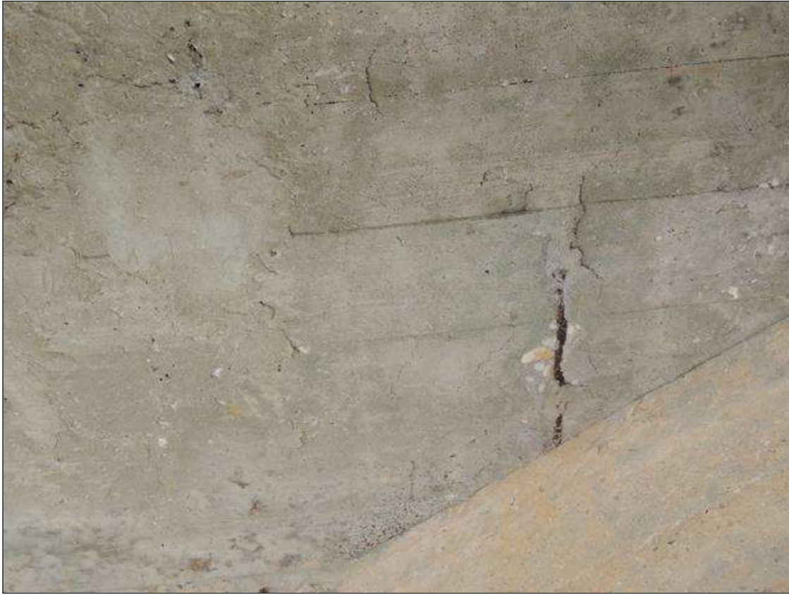
Span 2 Deck: 4 Square Feet of Delamination/Spall: Delaminated. Spall 1 in. or less deep or 6 in. or less in diameter. SPAN 2 BOTTOM OF DECK OF BAY 3 OVER BENT 1 CAP CRACKED AND DELAMINATED AREA WITH REBAR EXPOSED.
