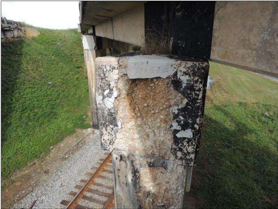
BT. 2 CAP LT. END, NORTH & SOUTH FACES HEAVLY CRACKED, DELAM, SPALLED & DETERIORATED. 3' N & S FACE 37" WIDE X 37" DOWN X 4" DEEP.
