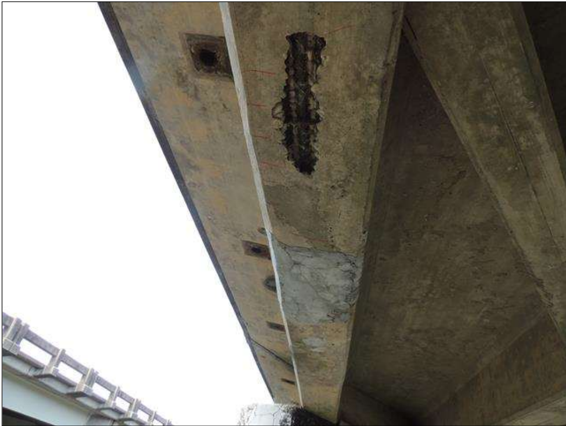
SP. 2 G1 FROM MIDSPAN NORTH 13'. LT., RT. FACES & BOTTOM SPALLED, CRACKED, DELAM. & PATCHED. SPALLED AREA 10" X 50" X 3 1/2" D.3 REBAR EXPOSED.
