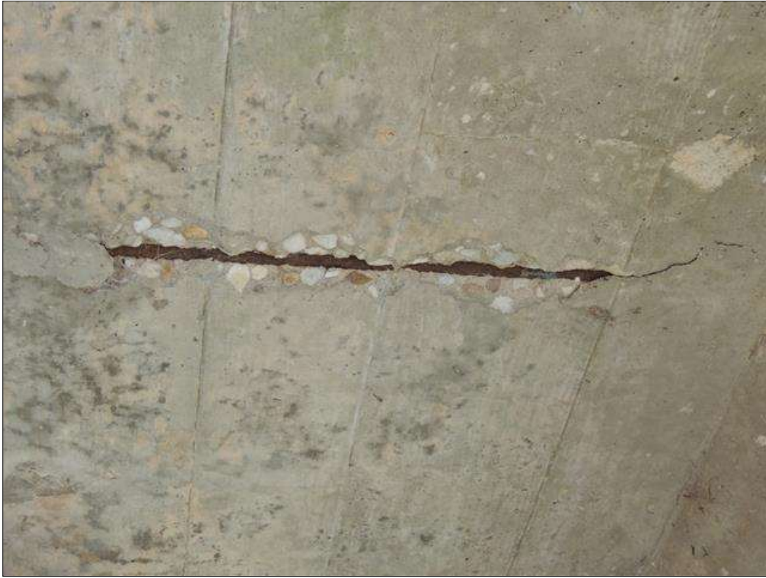
Span 4 Deck: 3 Square Feet of Delamination/Spall: Delaminated. Spall 1 in. or less deep or 6 in. or less in diameter. BOTTOM OF DECK BAY 2 NEAR BENT 4 HAS SURFACE SPALL AREA 4" WIDE X 24" LONG.
