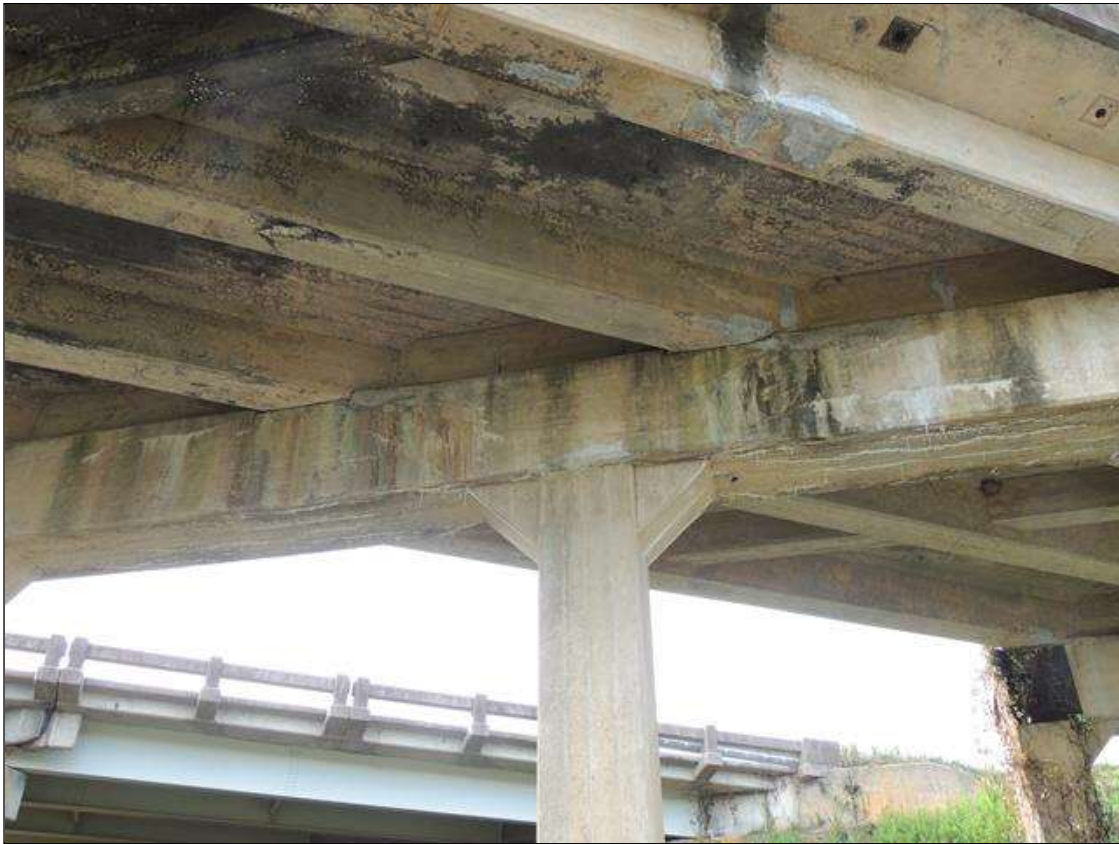
Bent 3 Cap : 8 Feet of Cracking (RC and Other): Width greater than 0.05 in. or spacing of less than 1 ft. SOUTH FACE OF CAP HAS MAP CRACKING WITH HEAVY EFFLO LEFT OF G 2 TO G 4.
