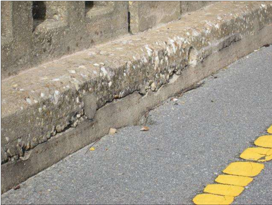
Span 2 Left Bridge Rail: 41 Feet of Cracking (RC and Other): Width 0.012-0.05 in. or spacing of 1.0-3.0 ft. LEFT CURB FACE IS CRACKED FULL LENGTH.
