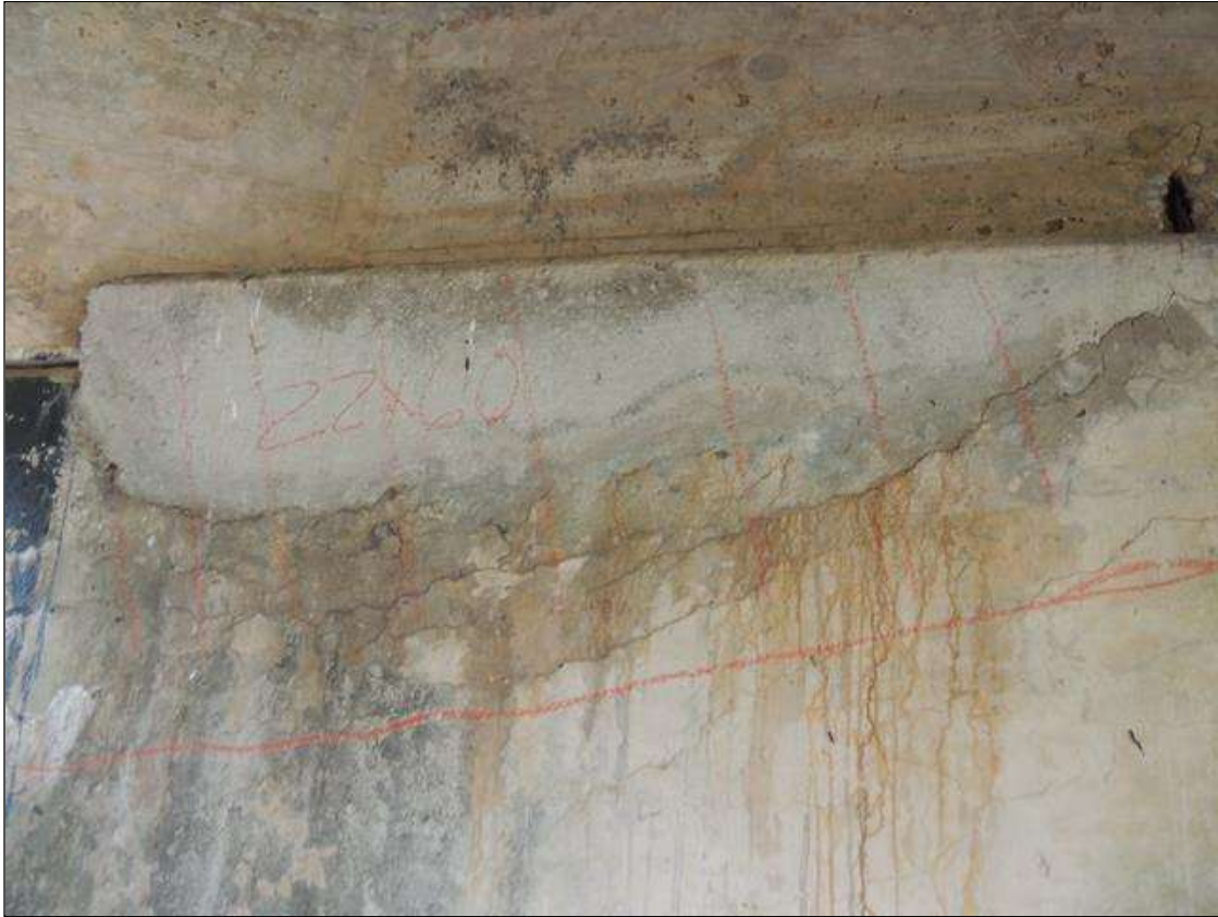
Bent 1 Cap : 5 Feet of Delamination/Spall/Patched Area: Delaminated. Spall 1 inch or less deep or 6 inches or less in diameter. Patched area that is sound BENT 1 SOUTH FACE OF CAP RIGHT SIDE OF G1 CRACKED AND PATCHED AREA IS DELAMINATED TOP DOWN 22" 5' LONG.
