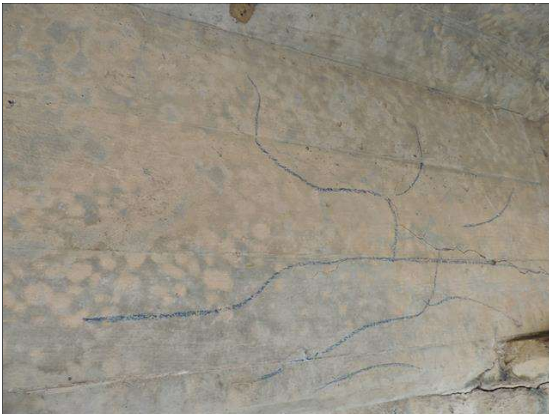
Span 4 Beam 2: 7 Feet of Cracking (RC and Other): Width 0.012-0.05 in. or spacing of 1.0-3.0 ft. RIGHT SIDE OF G 2 HAS SCATTERED MAP CRACKING AT BENT 4
