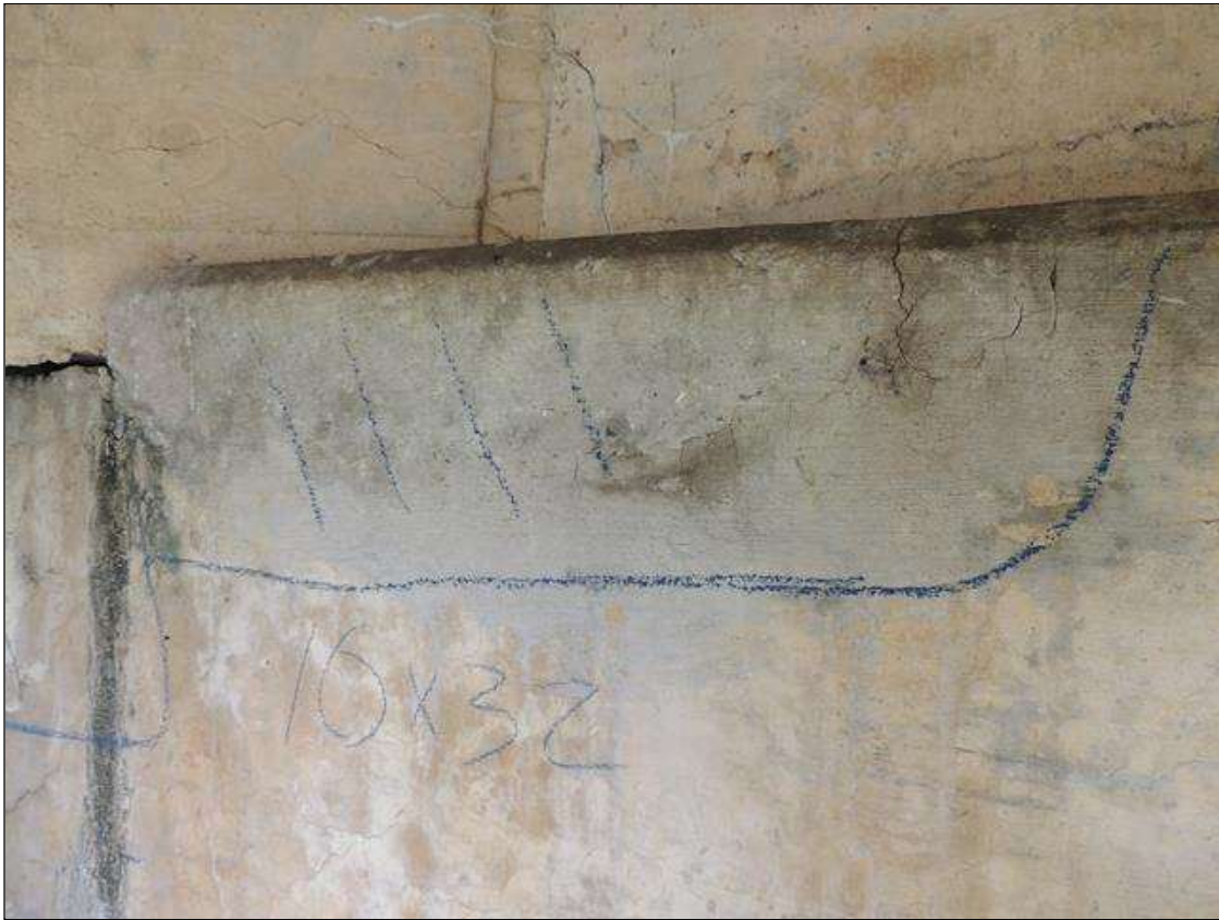
Bent 2 Cap : 3 Feet of Delamination/Spall/Patched Area: Delaminated. Spall 1 inch or less deep or 6 inches or less in diameter. Patched area that is sound BENT 2 SOUTH FACE OF CAP CRACKED AND DELAMINATED AND PATCHED AREA RIGHT SIDE OF G3 10" DOWN FACE AND 32" LONG.
