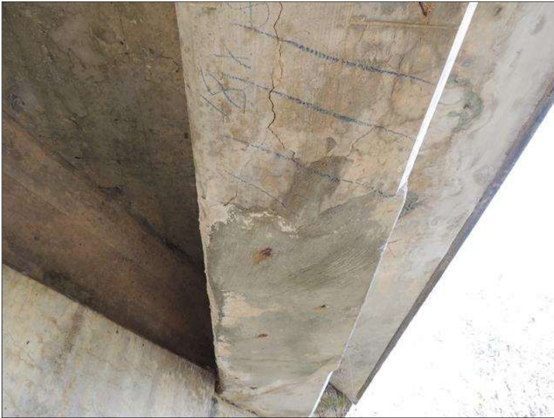
Span 4 Beam 4: 7 Feet of Delamination/Spall/Patched Area: Delaminated. Spall 1 in. or less deep or 6 in. or less in diameter. BOTTOM OF G 4 IS CRACKED, PATCHED AND DELAMINATED FROM BENT 4 BACK 7' 18" WIDE AND UP FACE 5".
