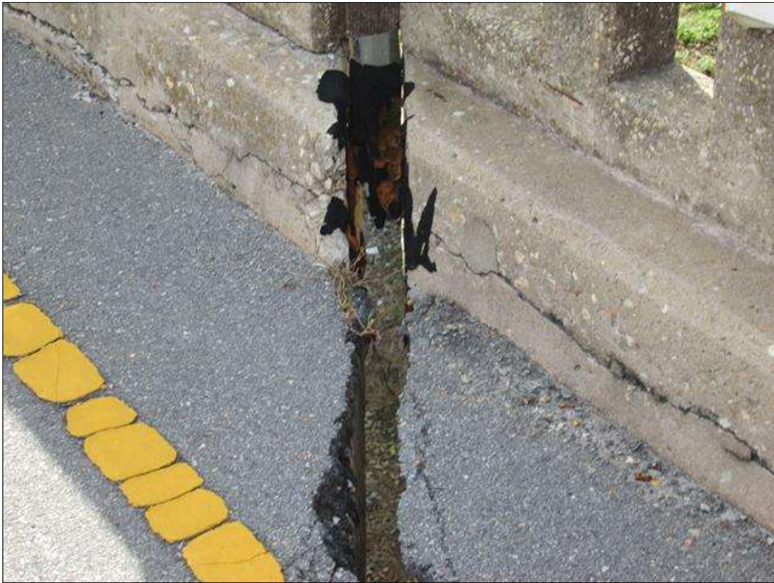
Expansion Joint 4 : 0 Feet of Leakage: Free flow of water through the joint. JOINT MATERIAL IS MISSING IN THE LEFT CURB AREA. THE OPENING IS 3" AND THE SPANS ARE MISALIGNED.
