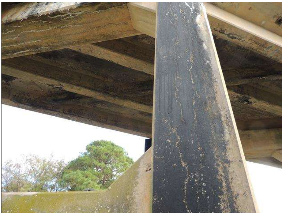
Bent 3 Pile 1: 0 Each of Cracking (RC and Other): Width 0.012-0.05 in. or spacing or 1.0-3.0 ft. NORTH FACE OF COL. HAS SCATTERED MAP AND VERTICAL CRACKS. SIMILAR ON THE EAST AND SOUTH FACES.
