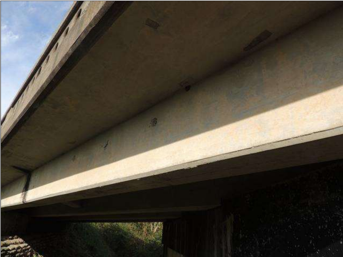
Span 5 Beam 1: 30 Feet of Cracking (RC and Other): Width 0.012-0.05 in. or spacing of 1.0-3.0 ft. LEFT SIDE OF G1 HAS SCATTERED MAP CRACKING IN FACE.
