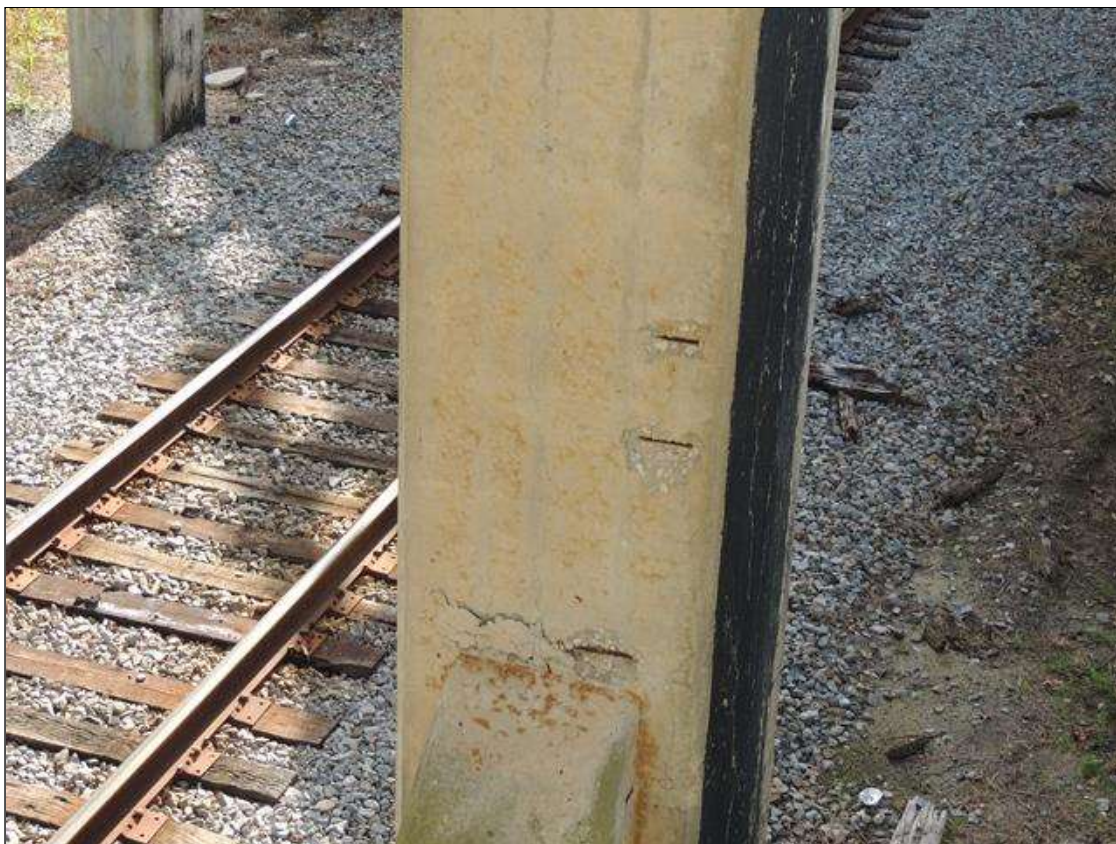
Bent 3 Pile 1: 1 Each of Delamination/Spall/Patched Area: Delaminated. Spall 1 in. or less deep or 6 in. or less in diameter. COL. 1 EAST FACE HAS 3 SPALLED AREAS ABOVE SRTUT. AREAS ARE 5" X 5" X 3/4" DEEP AND 7" X 18" X 3/4" DEEP.
