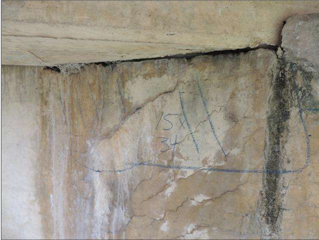
Bent 2 Cap : 3 Feet of Delamination/Spall/Patched Area: Delaminated. Spall 1 inch or less deep or 6 inches or less in diameter. Patched area that is sound BENT 2 SOUTH FACE OF CAP CRACKED AND DELAMINATED AREA WITH HEAVY EFFLO UNDER G3.
