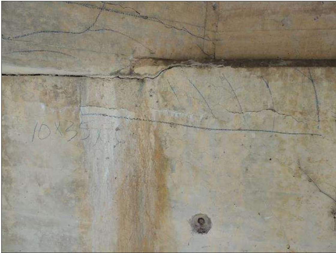
Bent 4 Cap : 3 Feet of Delamination/Spall/Patched Area: Delaminated. Spall 1 inch or less deep or 6 inches or less in diameter. SOUTH FACE OF CAP IS CRACKED AND DELAMINATED RIGHT OF G 2. AREA IS 10" DOWN FACE 35" LONG & 5" ON TOP.
