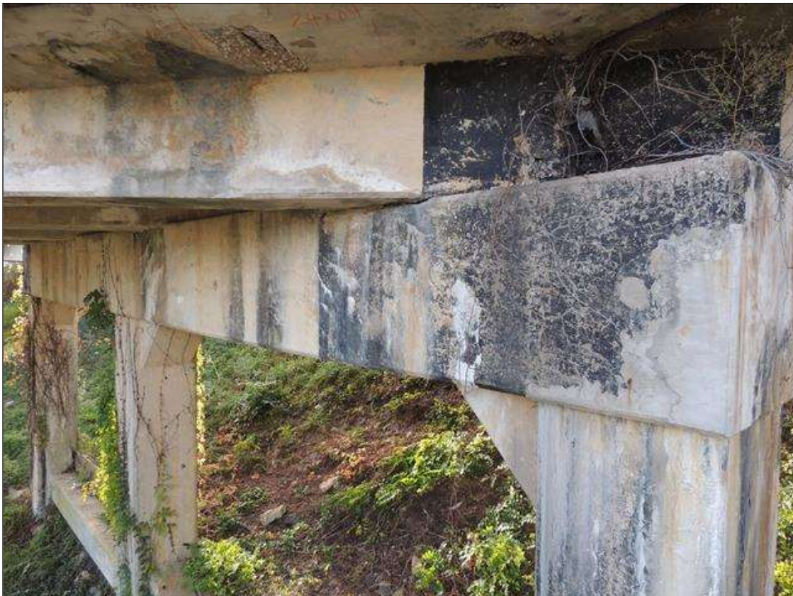
Bent 4 Cap : 0 Feet of Cracking (RC and Other): Width 0.012-0.05 in. or spacing of 1.0-3.0 ft. SOUTH FACE OF CAP HAS SCATTERED MAP CRACKING WITH EFFLO STAINING.
