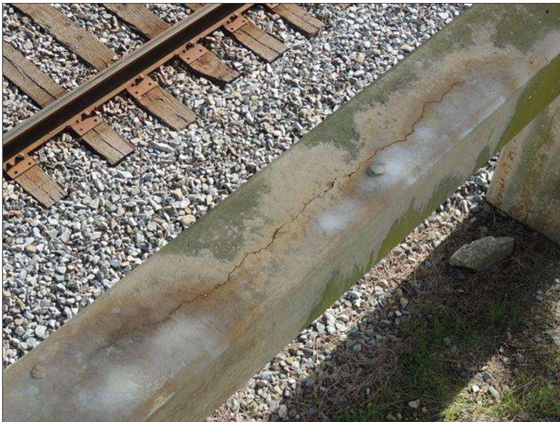
TOP OF STRUT BETWEEN COL. 1 AND COL. 2 @ BENT 3 IS CRACKED ON TOP 12' LONG
