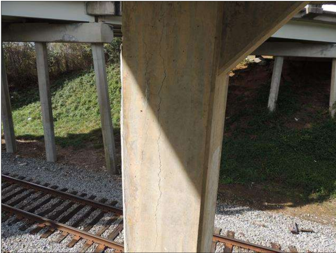
Bent 2 Pile 1: 0 Each of Cracking (RC and Other): Width 0.012-0.05 in. or spacing or 1.0-3.0 ft. BENT 2 COL 1 SOUTH FACE OF CAP VERTICAL AND MAP CRACKING FROM TOP TO BOTTOM AND ALL OTHER FACES ARE SIMILAR.
