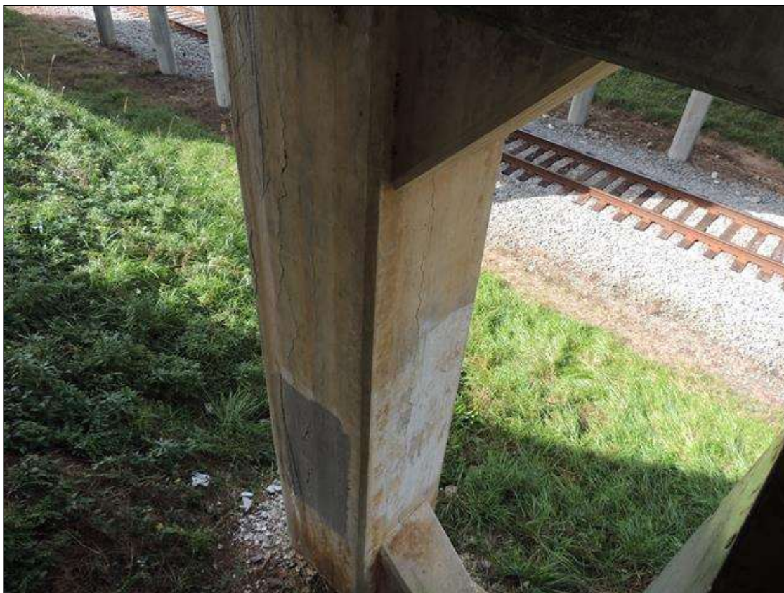
Bent 1 Pile 1: 0 Each of Cracking (RC and Other): Width 0.012-0.05 in. or spacing or 1.0-3.0 ft. BENT 1 COL 1 SOUTH AND EAST FACE OF COL HEAVY VERTICAL AND MAP CRACKING AND NORTH FACE IS SIMILAR.
