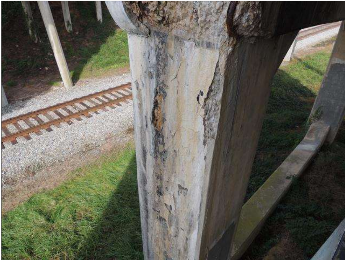
BT. 1 COL. 1 WEST FACE CRAKED, DELAM. & DETERIORATED. TOP TO BOTTOM 13' X 31" WIDE WITH HEAVY EFFLO AND EXTENDS AROUND SOUTH & NORTH FACES 10"
