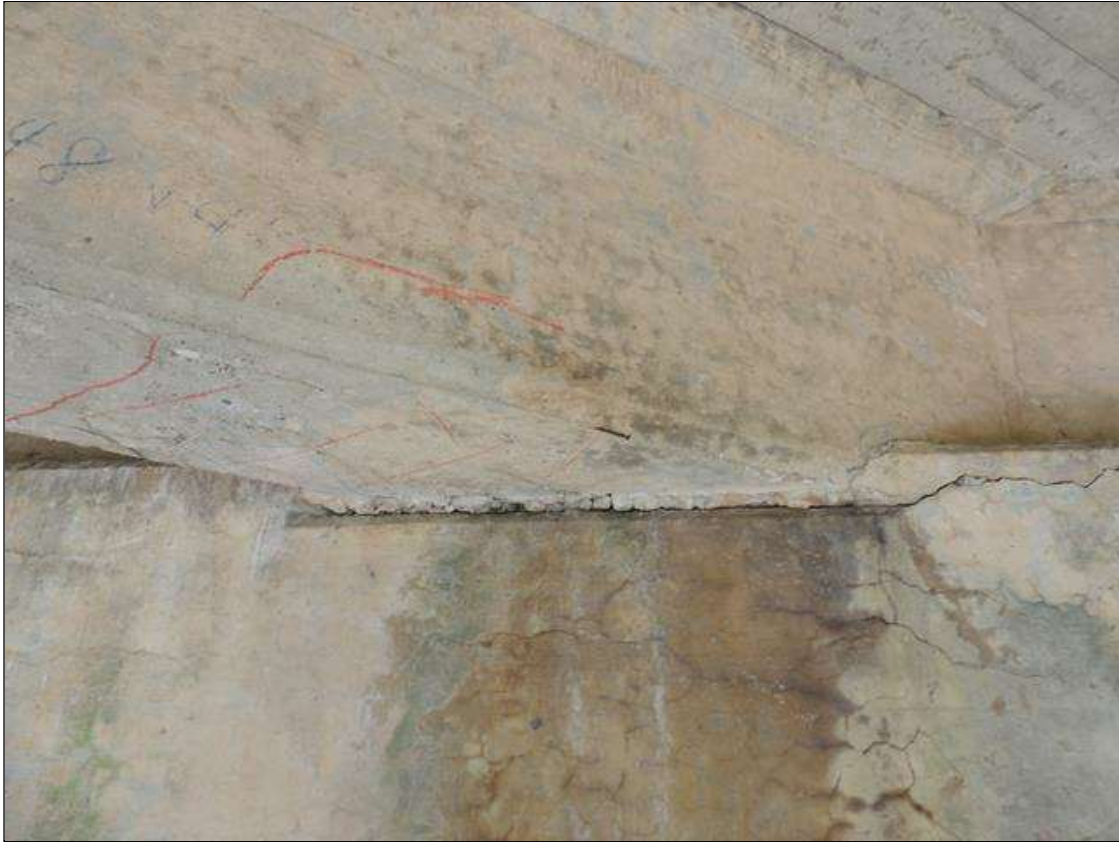
Span 2 Beam 3: 4 Feet of Delamination/Spall/Patched Area: Delaminated. Spall 1 in. or less deep or 6 in. or less in diameter. Patched area that is sound. SPAN 2 LEFT AND RIGHT SIDE OF G3 AND BOTTOM CRACKED AND DELAMINATED FROM END OF GIRDER OVER BENT 1 OUT 4' 18" UNDER BOTTOM AND 4" UP THE FACE.
