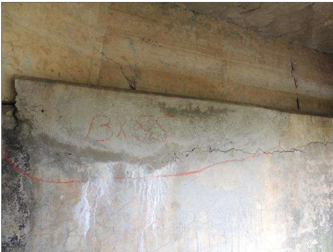
Bent 1 Cap : 5 Feet of Delamination/Spall/Patched Area: Delaminated. Spall 1 inch or less deep or 6 inches or less in diameter. Patched area that is sound BENT 1 SOUTH FACE OF CAP HAS A PATCHED AREA ALONG TOP FACE RIGHT SIDE OF G3 13" DOWN FACE AND 55 " LONG.
