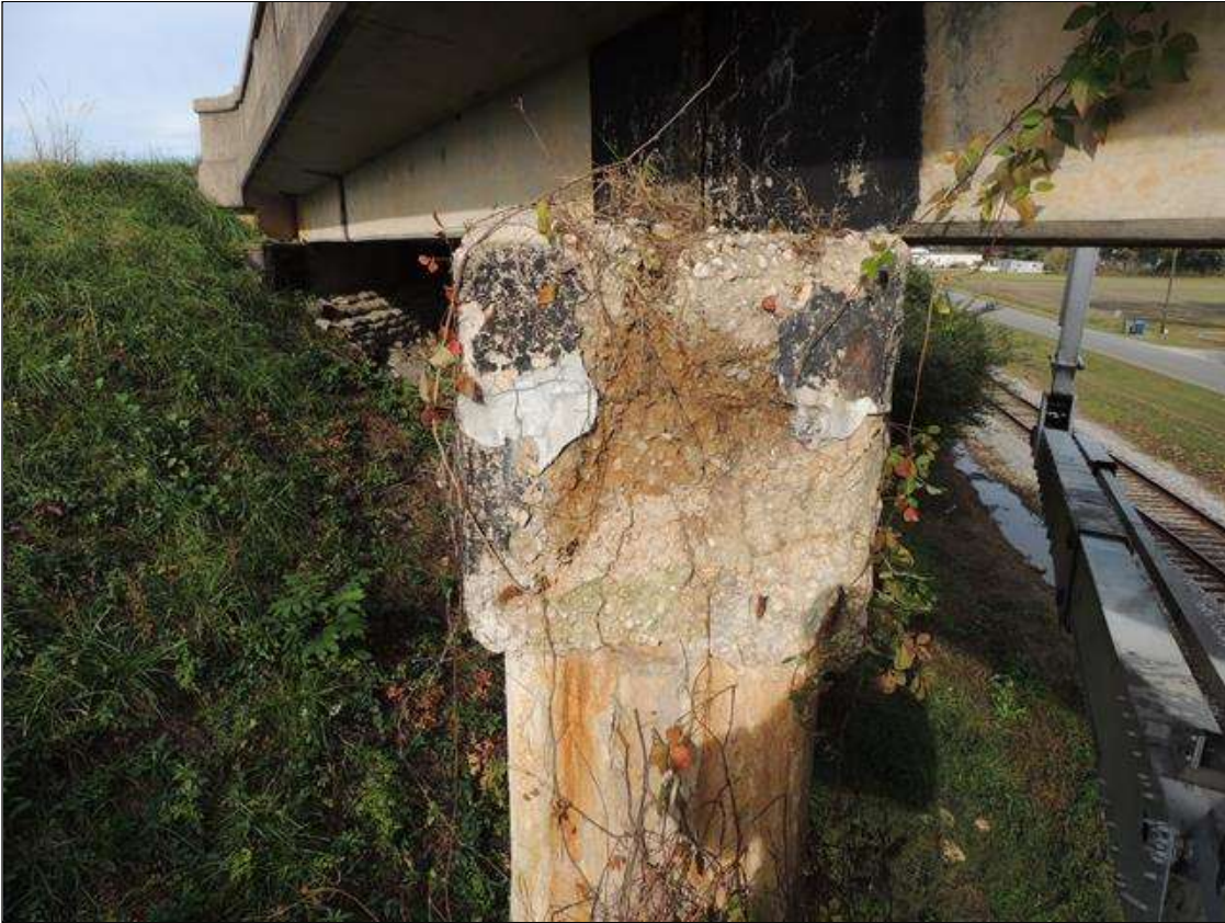
Bent 4 Cap : 6 Feet of Delamination/Spall/Patched Area: The condition warrants structural review to determine the effect on strength and serviceability of the element or the bridge; OR a structural review has been completed and the defects impact strength or serviceability of the element or bridge. LEFT END OF CAP IS SPALLED & DELAMINATED. 3' ON SOUTH AND NORTH FACES. 37" X 37" ON END UP TO 4" DEEP.
