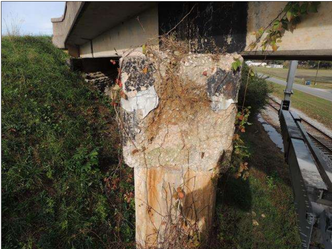
BT. 4 LT. END OF CAP CRACKED, SPALLED, DELAM. & DETERIORATED 3' ON N & S FACE AND 37" X 37" ON END 3" TO 4" DEEP.
