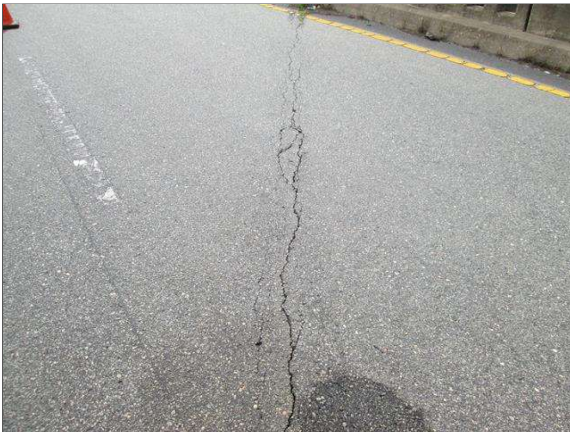
Expansion Joint 3 : 42 Feet of Seal Cracking: Surface crack. ASPHALT OVER BENT 2 IS CRACKED.
