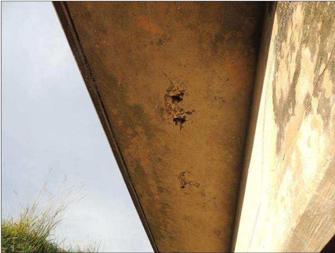
Span 5 Deck: 2 Square Feet of Delamination/Spall: Delaminated. Spall 1 in. or less deep or 6 in. or less in diameter. THE LEFT OVERHANG BOTTOM OF DECK HAS TWO AREAS SPALLED AND DELAMINATED 15' FROM END BENT 2. ONE AREA IS 6" X 10" AND 7" X 12".
