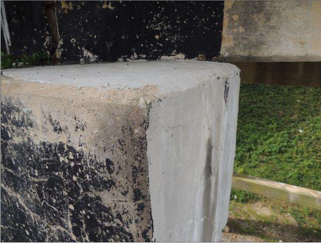
BENT 2 TOP OF CAP AND RIGHT END OF CAP HAS CONCRETE SMOOTH ON TOP AND END AND IS MAP CRACKED ON SOUTH RIGHT END AND NORTH FACES.
