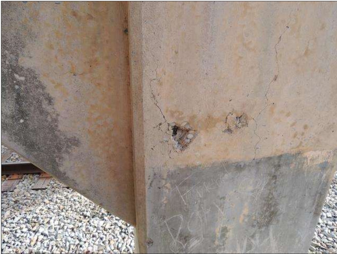
Bent 3 Pile 2: 1 Each of Delamination/Spall/Patched Area: Delaminated. Spall 1 in. or less deep or 6 in. or less in diameter. COL. HAS CRACKED , SPALLED AND DELAMINATED AREAS 6' ABOVE GROUND 7" X 12".
