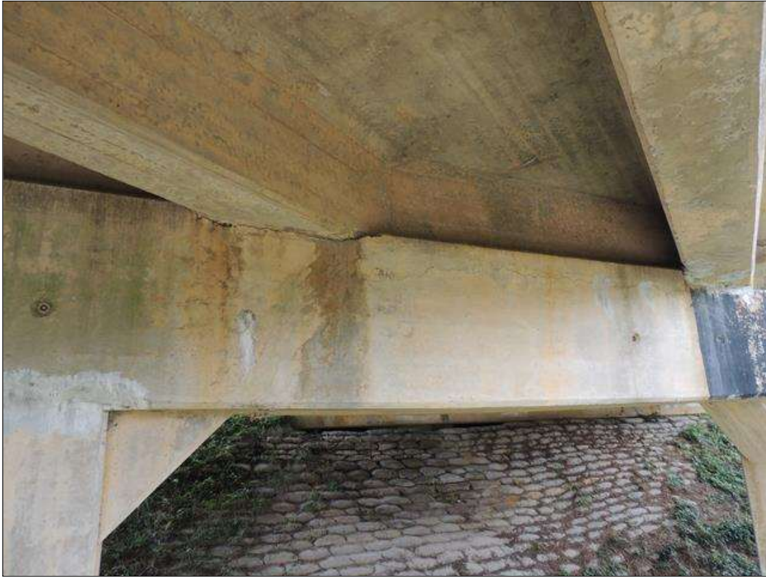
Bent 1 Cap : 0 Feet of Cracking (RC and Other): Width 0.012-0.05 in. or spacing of 1.0-3.0 ft. BENT 1 NORTH FACE OF CAP SCATTERED MAP CRACKING AND HORIZ CRACKS FROM LEFT TO RIGHT END.
