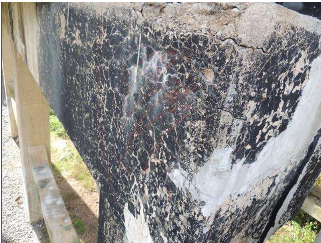
Bent 3 Cap : 3 Feet of Delamination/Spall/Patched Area: Spall greater than 1 inch deep or greater than 6 inches in diameter. SOUTH FACE OF CAP @ RIGHT END HAS A AREA THAT IS CRACKED SPALLED AND DELAMINATED. THE AREA IS 30" X 36".
