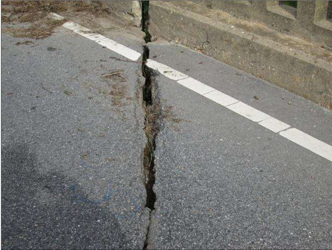
Expansion Joint 5 : 8 Feet of Leakage: Moderate. More than a drip and less than free flow of water. JOINT MATERIAL IS MISSING IN RIGHT LANE FROM RIGHT CURB OUT 8'. THIS AREA HAS SOME DEBRIS.
