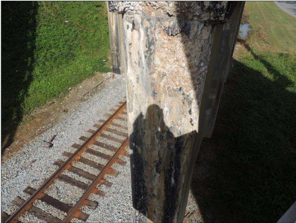
BT. 2 COL.1 W FACE CRACKED, DELAM, SPALLED & DETERIORATED WITH EFFLO. FROM BOTTOM OF CAP DOWN 20' X 30" W X 9" ON EACH FACE 3" DEEP.
