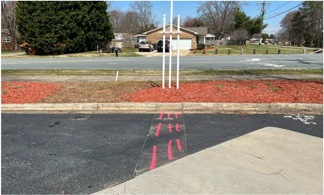
Photograph 5. Vent line at Shell Station property.
