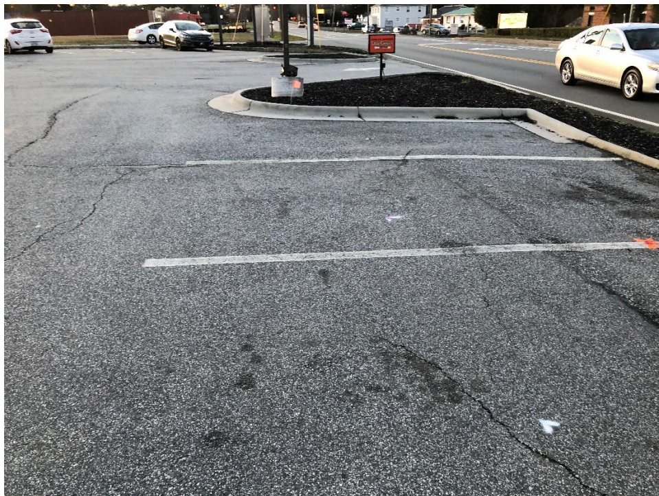
Photo 16: Looking north along Old Hollow Rd. showing asphalt cracking.
