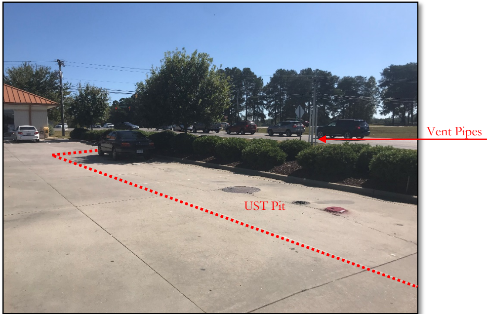
Photograph No. 1: General view of the Rushco UST Pit and Vent Pipes.
