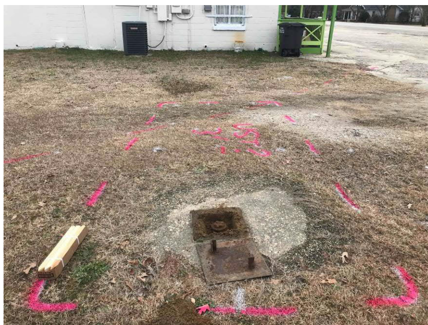
Photo #4 View of a typical exposed fill port for the on-site probable USTs; facing southeast.
