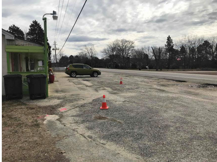
Photo #5 View of the possible fuel line extending from the probable USTs to western side of the on-site building; facing southeast.
