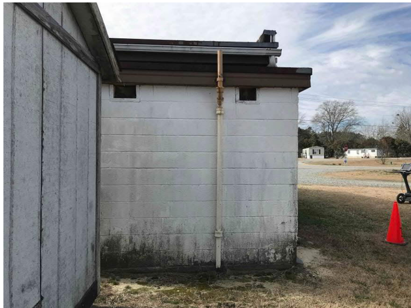
Photo #6 View of a vent pipe attached to eastern wall of the on-site building; facing west.
