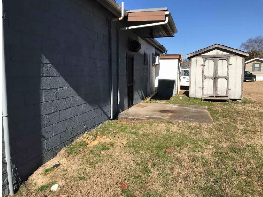
Photo #5 View of the eastern side of the on-site building and the underground sanitary sewer line located using a radiodetection pipe locator and marked with pink dots; facing north.
