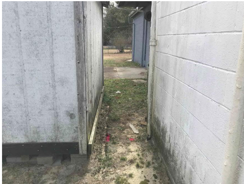
Photo #8 View of the apparent direction of vent pipes located using a radiodetection pipe locator; facing south.
