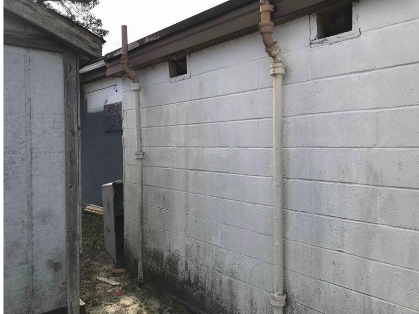
Photo #7 View of two vent pipes attached to eastern wall of the on-site building; facing south.
