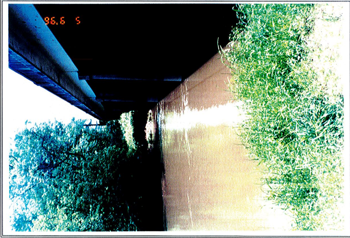
PHOTO NO. 5 - View of east side of the bridge, looking south showing locations of the water borings SBLB1-B, SBLB2-B, NBLB1-A, NBLB2-A, NBLB1-B, and NBLB2-B
