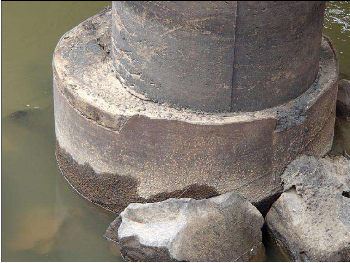
TYPICAL SURFACE RUST AND SCALE ON STEEL CASINGS
