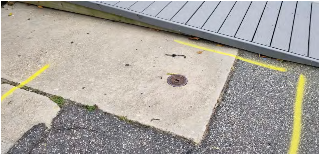
Photograph 4. Parcel 006 fill port on probable UST 4.
