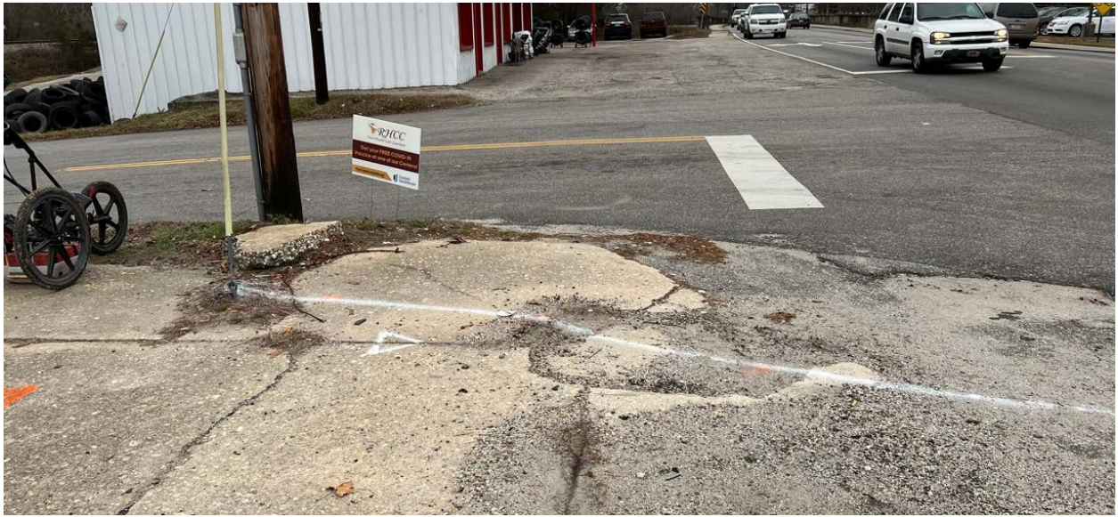
Photograph 3. Suspected unknown utility identified with white ground-marking paint.
