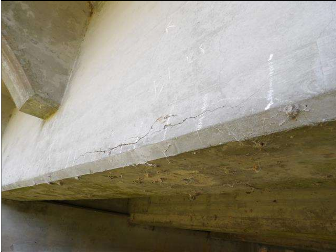
Span 2 Beam 5: 9' FROM BENT 1. 2' LONG X 5" HIGH AREA OF DELAMINATION WITH ASSOCIATED CRACKING IN RIGHT BOTTOM FACE
