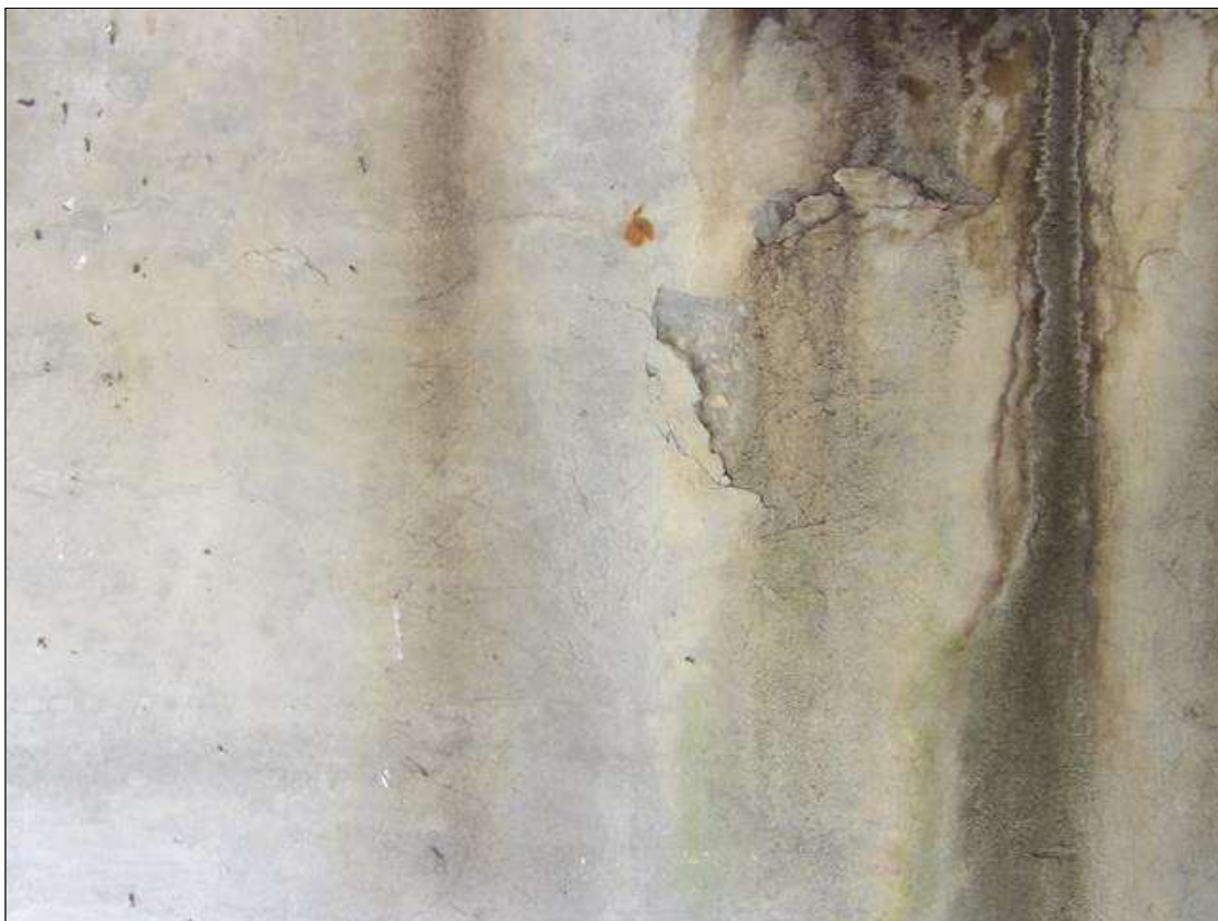
Bent 4 Cap 1: 3' LONG X 1.5' AREA OF DELMINATION WITH DETERIORATING CONCRETE IN EAST FACE BELOW BEAM 4
