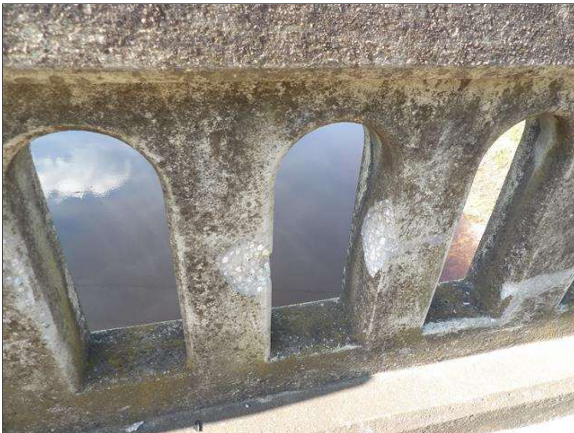
Span 3 Right Bridge Rail: 2 SPALLS LOCATED 6' BEFORE BENT 3, 4" DIAMETER EACH UP TO 1" DEEP
