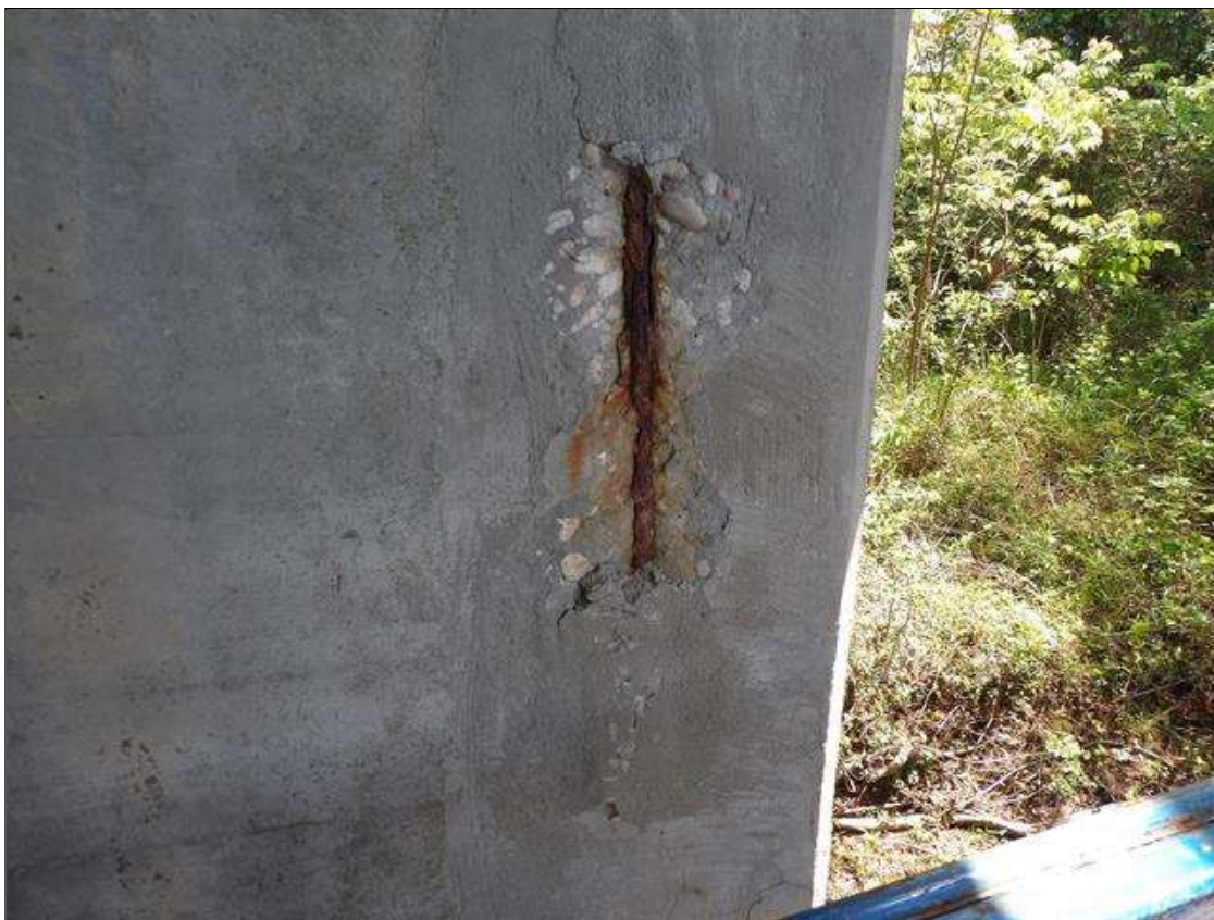
Bent 5 Cap 1: PAR -- 8" LONG X 15" HIGH X 1" DEEP SPALL WITH EXPOSED REBAR WITH MINOR SECTION LOSS ON WEST FACE AT PILE 8
