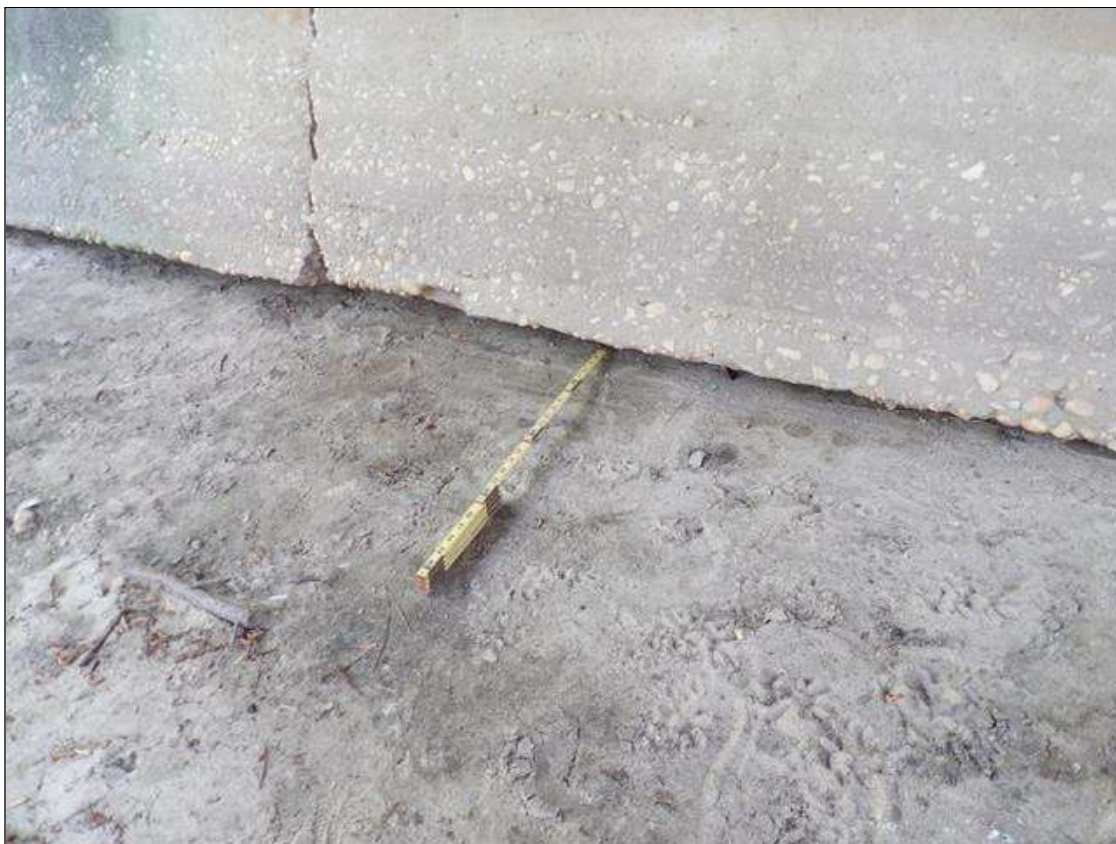
PAR -- 10' X 5" HIGH X 9" DEEP WASHOUT AND UNDERMINING OF THE SLOPE PROTECTION AT ABUTMENT 2
