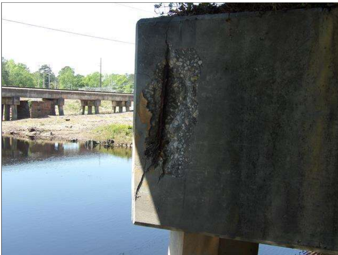
Bent 4 Cap 1: PAR -- SPALL 36" HIGH X 16" WIDE X 2.5" DEEP SPALL WITH EXPOSED REBAR WITH MINOR SECTION LOSS
