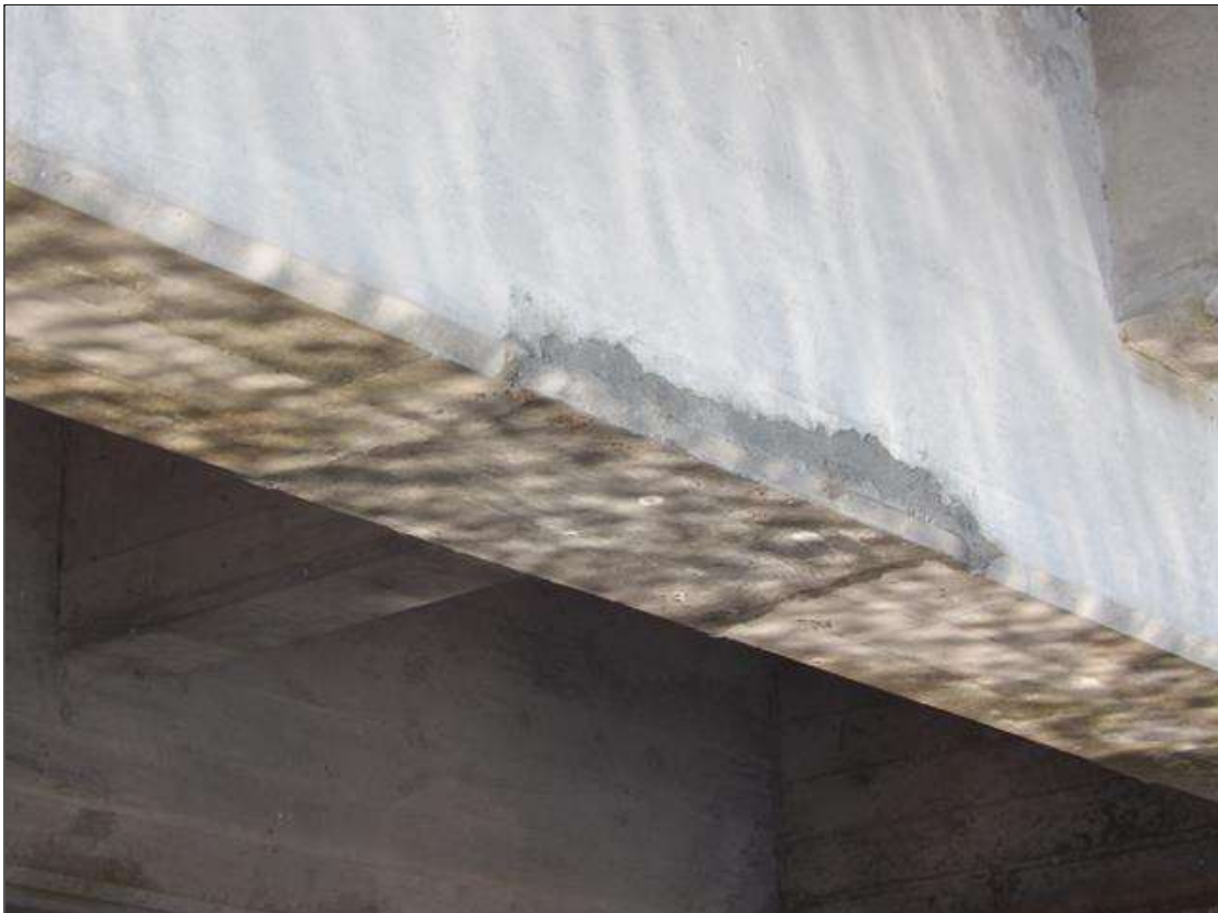
Span 4 Beam 5: 2.5' LONG X FULL WIDTH OF BOTTOM FLANGE AND EXTENDING 4" ON BOTH FACES SOUND PATCHED AREA 10' FROM BEANT 4
