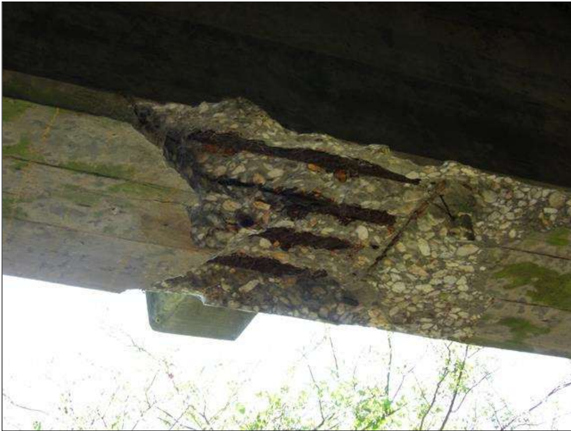
Span 6 Beam 5: PAR -- 20" LONG X FULL BOTTOM WIDTH X 3" DEEP SPALL WITH EXPOSED REBAR WITH MINOR SECTION LOSS IN BOTTOM OF FLANGE 10' FROM BENT 6
