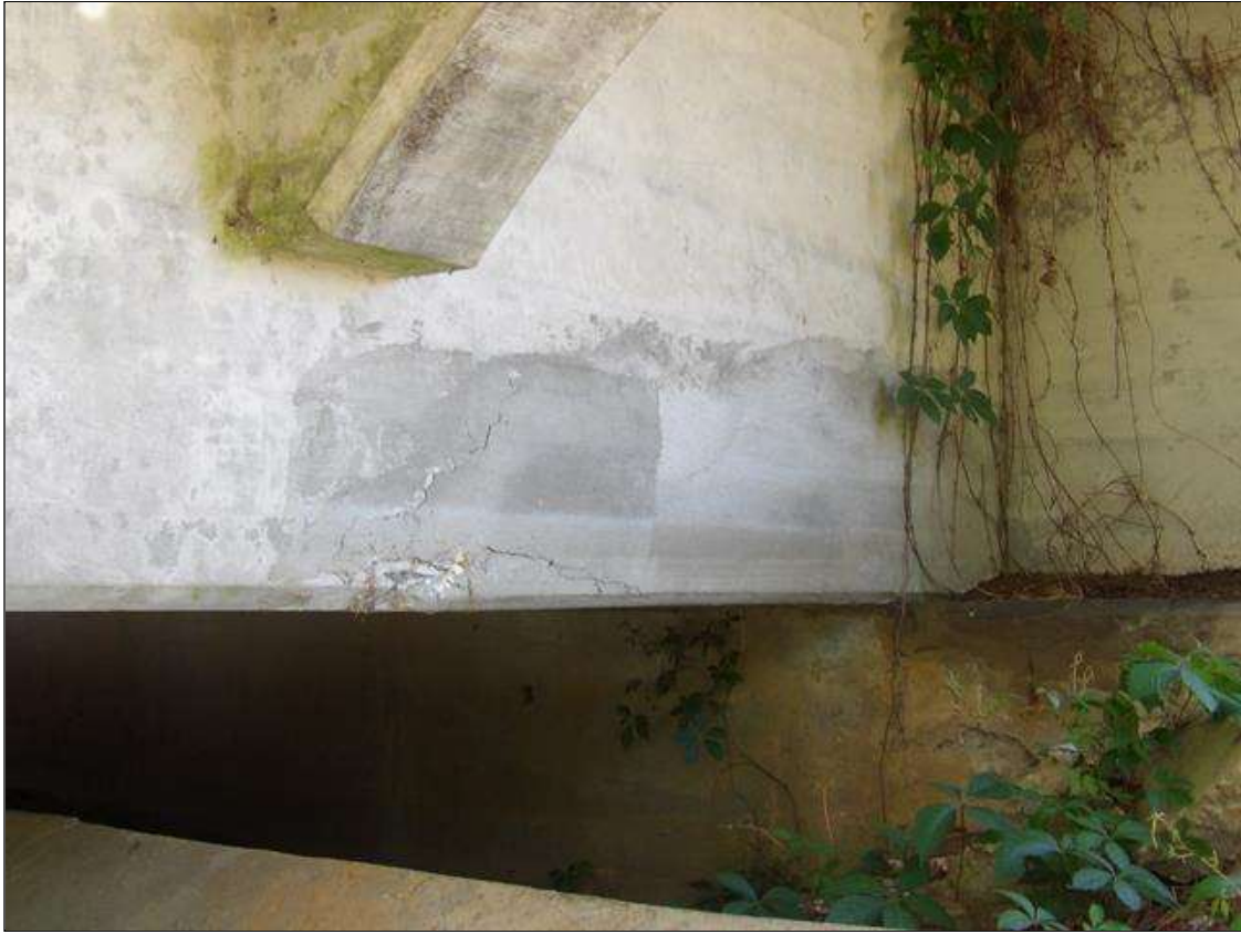
Span 1 Beam 1: LARGE FAILING PATCH 15' LONG X 2' WIDE ON LEFT BOTTOM FACE 18" FROM END BENT 1
