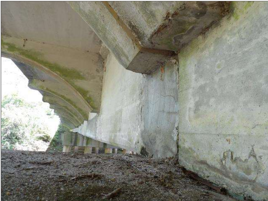
Span 4 Beam 1: 1' HIGH X 1' WIDE SOUND PATCHED AREA AT BENT 3 WITH HAIRLINE HORIZONTAL CRACKING
