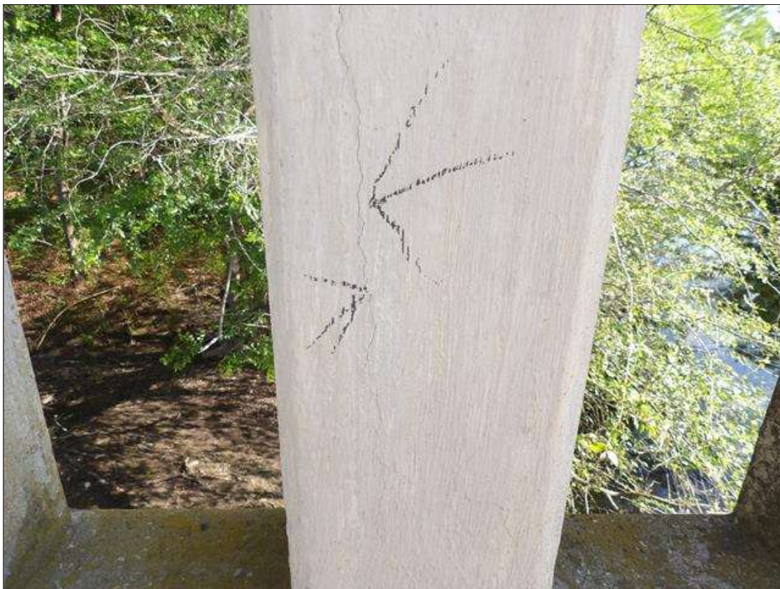
Span 3 Left Bridge Rail: HAIRLINE CRACKS IN LEFT RAIL POSTS AT VARIOUS LOCATIONS THROUGHOUT
