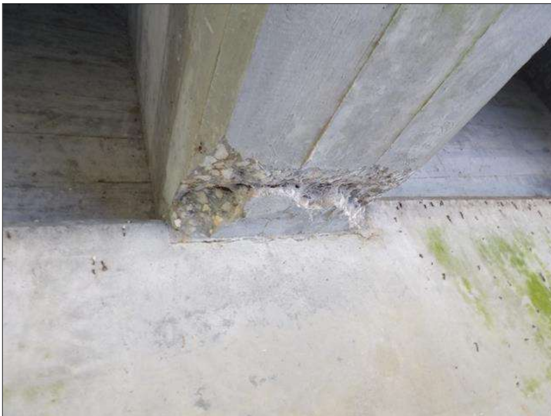
Span 4 Beam 3: 8" LONG X FULL WIDTH X 2" DEEP SPALL WITH NO EXPOSED REBAR IN BOTTOM FLANGE AT BENT 4
