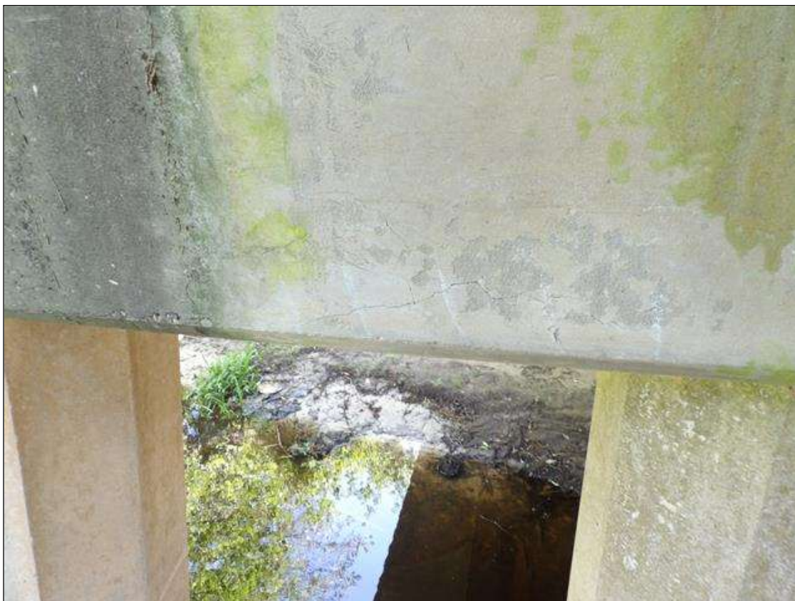
Bent 5 Cap 1: (2) 18" LONG X 15" WIDE AREA OF DELAMINATIONS ON THE WEST FACE AT BOTH ENDS OF CAP LEFT END SHOWN
