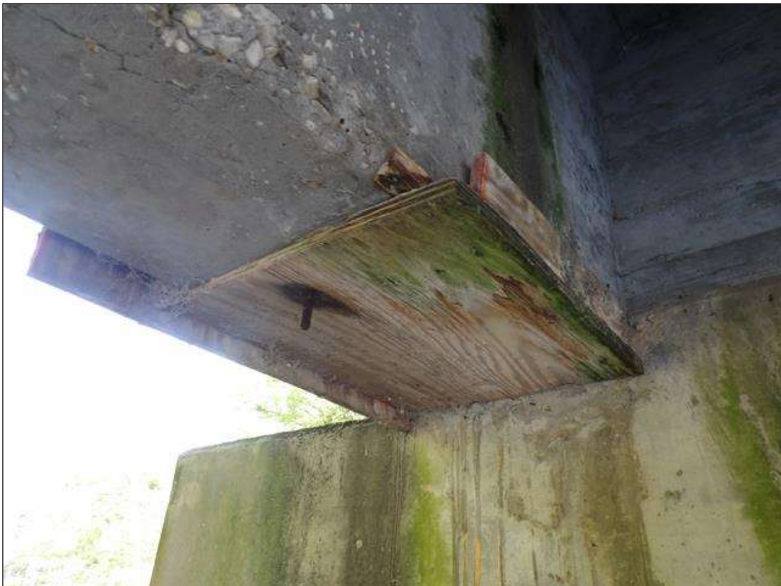
Span 4 Beam 1: CONSTRUCTION FORMS LEFT IN PLACE
