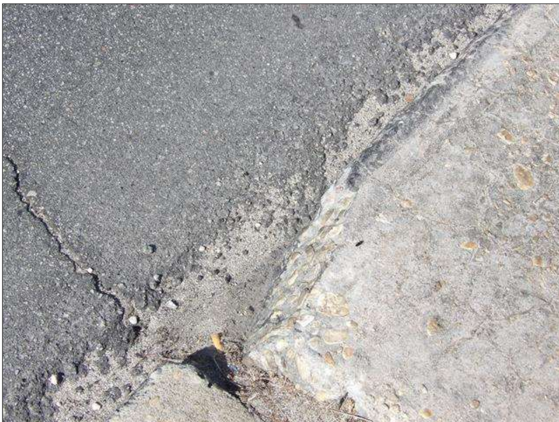
SIDEWALK AT EAST END, OVER END BENT 2, CORNER SPALL 8" X 6" X 1" DEEP
