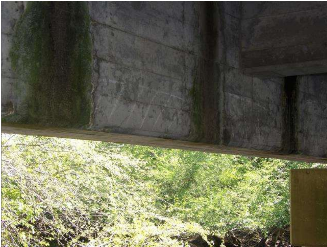
Span 3 Beam 1: 25' LONG X 8" WIDE ON BOTTOM FACE AND EXTENDING UP TO 2' HIGH ON WEB AREA OF DELAMINATION IN RIGHT FACE STARTING 4' FROM PIER 3
