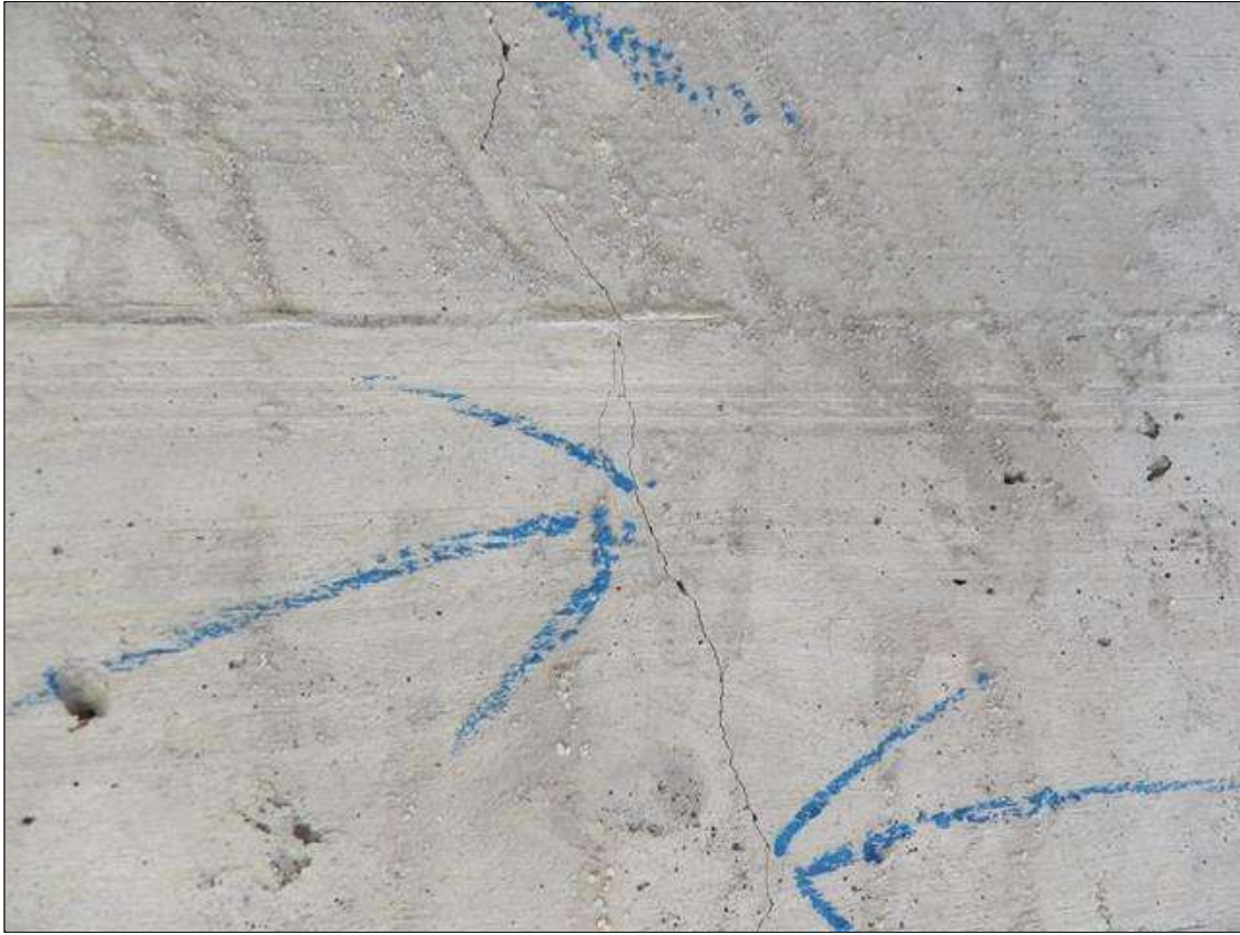
TYPICAL HAIRLINE VERTICAL CRACKS IN THE WEB AREA THROUGHOUT THE LENGTH OF THE BEAMS, SPAN 1 BEAM 5 SHOWN.
