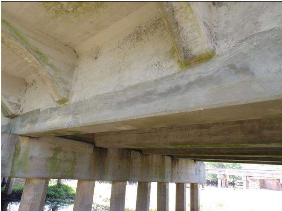
Span 1 Beam 1: 12' FROM BENT 1. FAILING PATCH 8' LONG X FULL BEAM WIDTH ON THE BOTTOM OF THE BEAM AND BOTH FACES.
