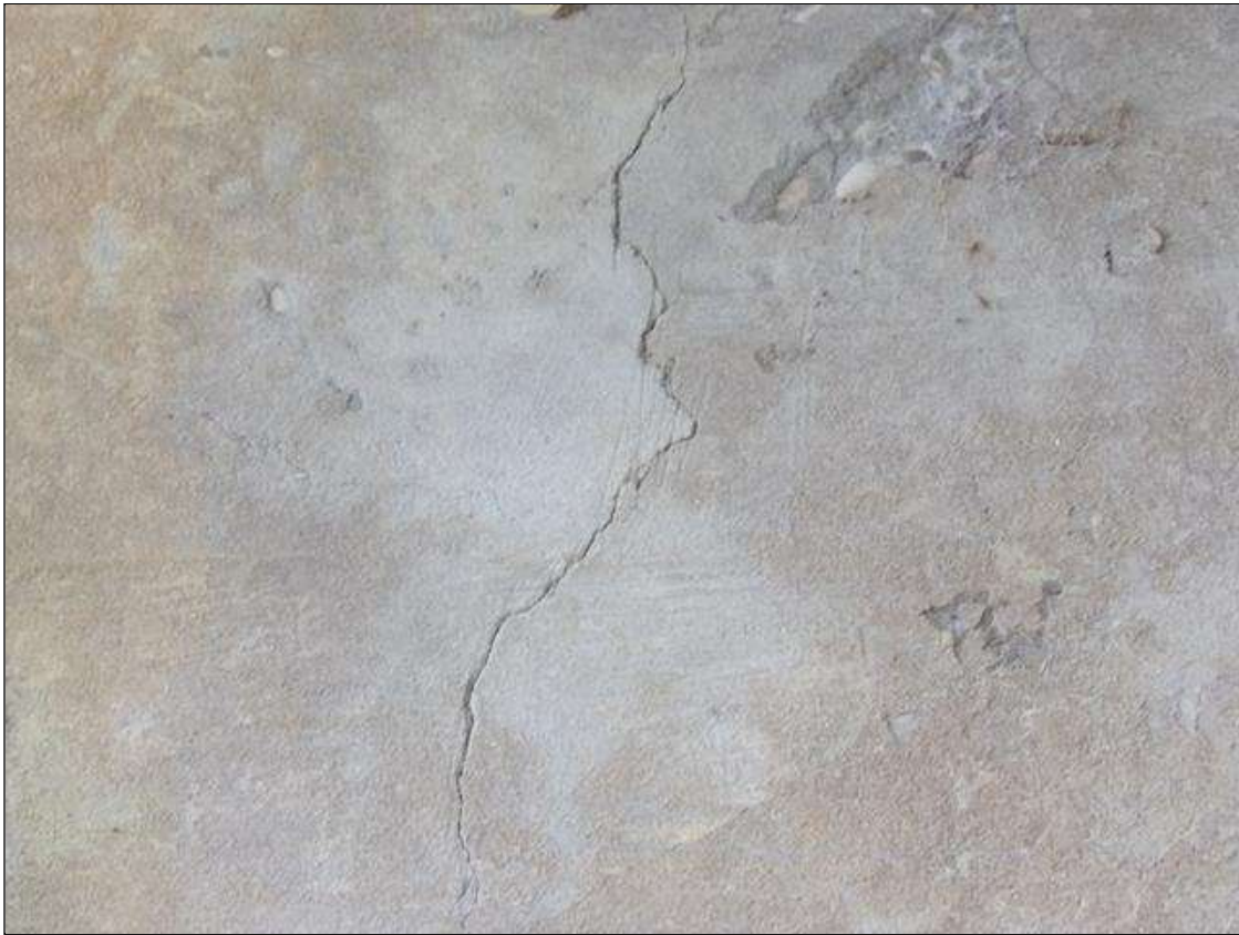
Bent 2 Cap 1: UP TO 1/32" WIDE VERTICAL AND DIAGONAL CRACKS UP TO 2' LONG THROUGHOUT BOTH FACES
