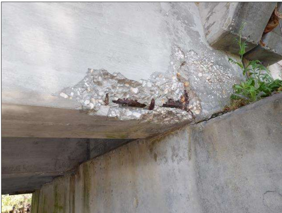
Span 4 Beam 5: PAR --- 2' LONG X UP TO 1' HIGH X 3" DEEP SPALL WITH EXPOSED REBAR WITH MINOR SECTION LOSS IN RIGHT FACE FACE OF WEB AT BENT 4
