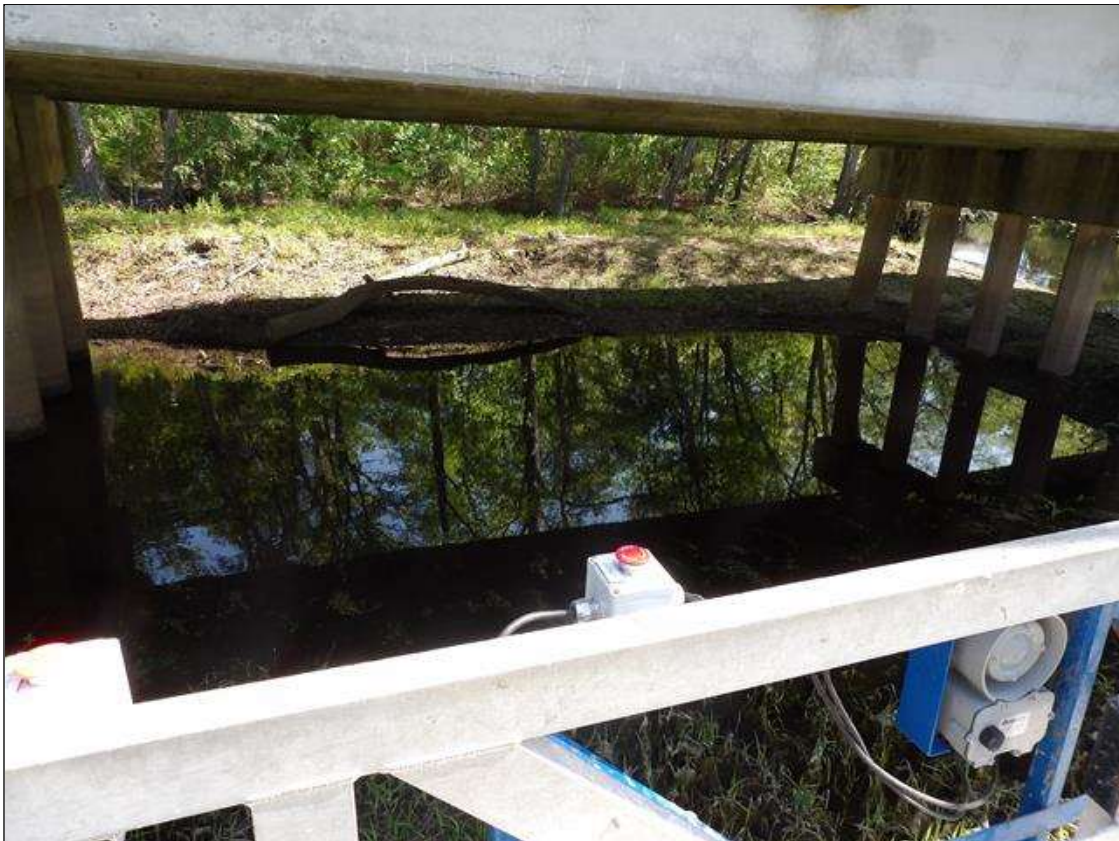
SPAN 2 FULL LENGTH X FULL WIDTH X 2' DEEP SCOUR HOLE WITH STANDING WATER
