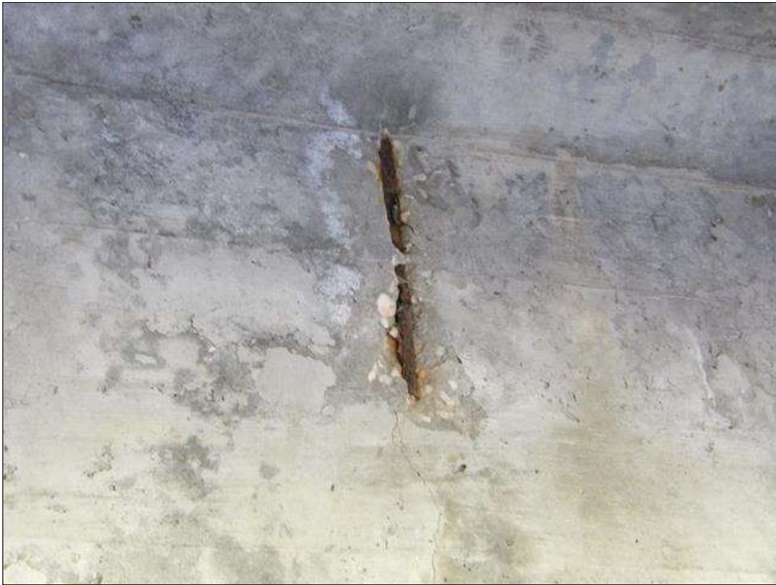
Span 2 Beam 1: 1' LONG X 3" WIDE X 1" DEEP SPALL WITH EXPOSED REBAR WITH NO MEASURABLE SECTION LOSS IN RIGHT FACE NEAR MIDSPAN
