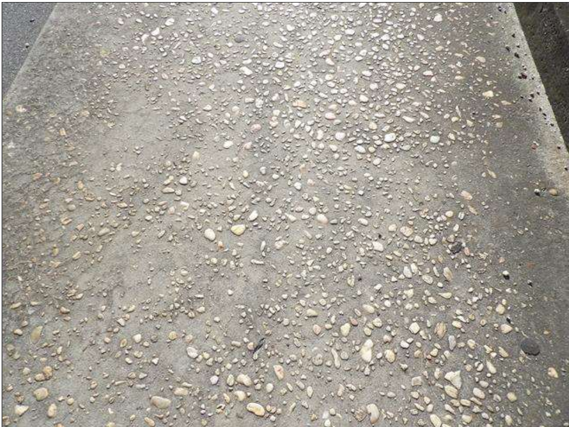
Typical minor abrasion on sidewalks, Span 1 right sidewalk shown
