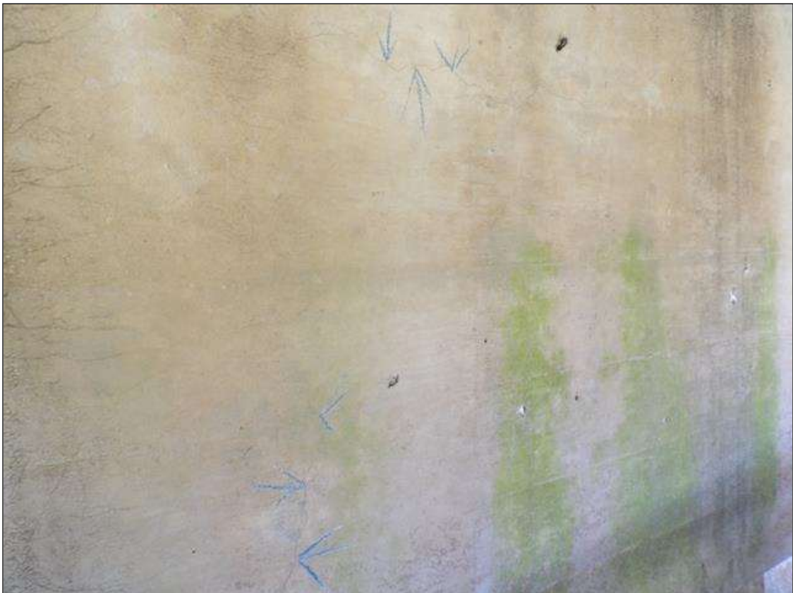
TYPICAL HAIRLINE TO 1/32" VERTICAL/HORIZONTAL CRACKS IN CAP, BENT 1 CAP SHOWN
