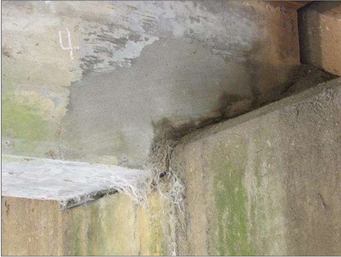
Span 4 Beam 3: 1' LONG X 10" HIGH SOUND PATCHED AREA IN LEFT FACE OF WEB AT BENT 3
