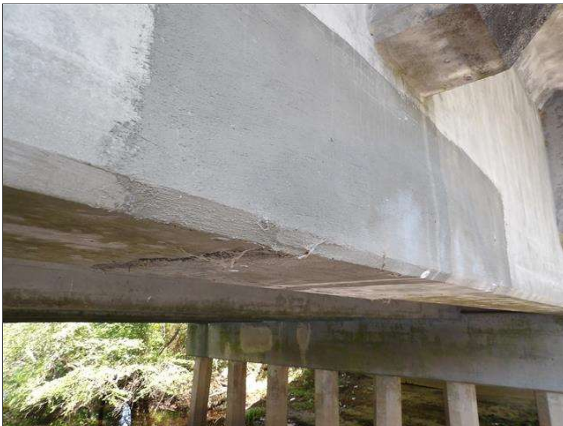
Span 5 Beam 5: 2.5' LONG X FULL WIDTH OF BOTTOM FLANGE SOUND PATCH AREA EXTENDING UP TO 1' ON BOTH FACES OF WEB, NEAR MIDSPAN
