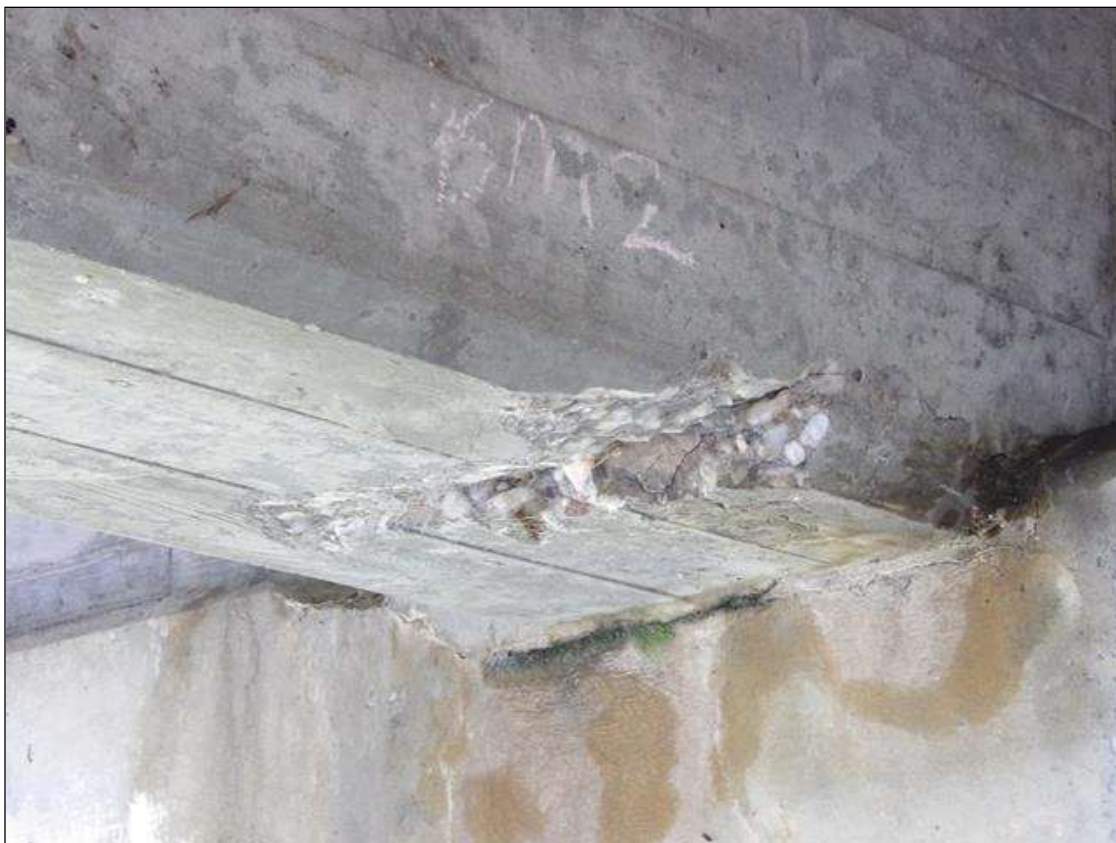
Span 3 Beam 4: 1' LONG X 8" WIDE X 2" DEEP SPALL IN BOTTOM FACE AT BENT 2
