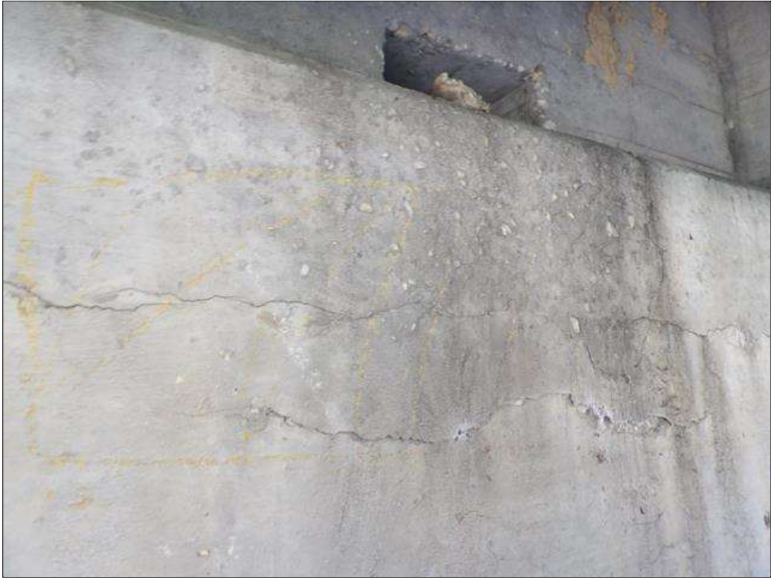
Bent 1 Cap 1: 5' LONG X 12" HIGH AREA OF DELAMINATION ON WEST FACE IN BAY 2
