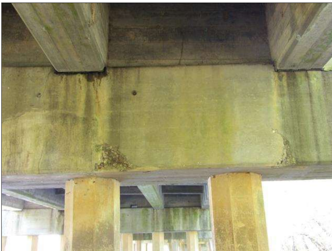
Bent 5 Cap 1: (2) UP TO 12" HIGH X 12" LONG X 3" DEEP SPALLS WITH NO EXPOSED REBAR ON EAST FACE UNDER BAY 1
