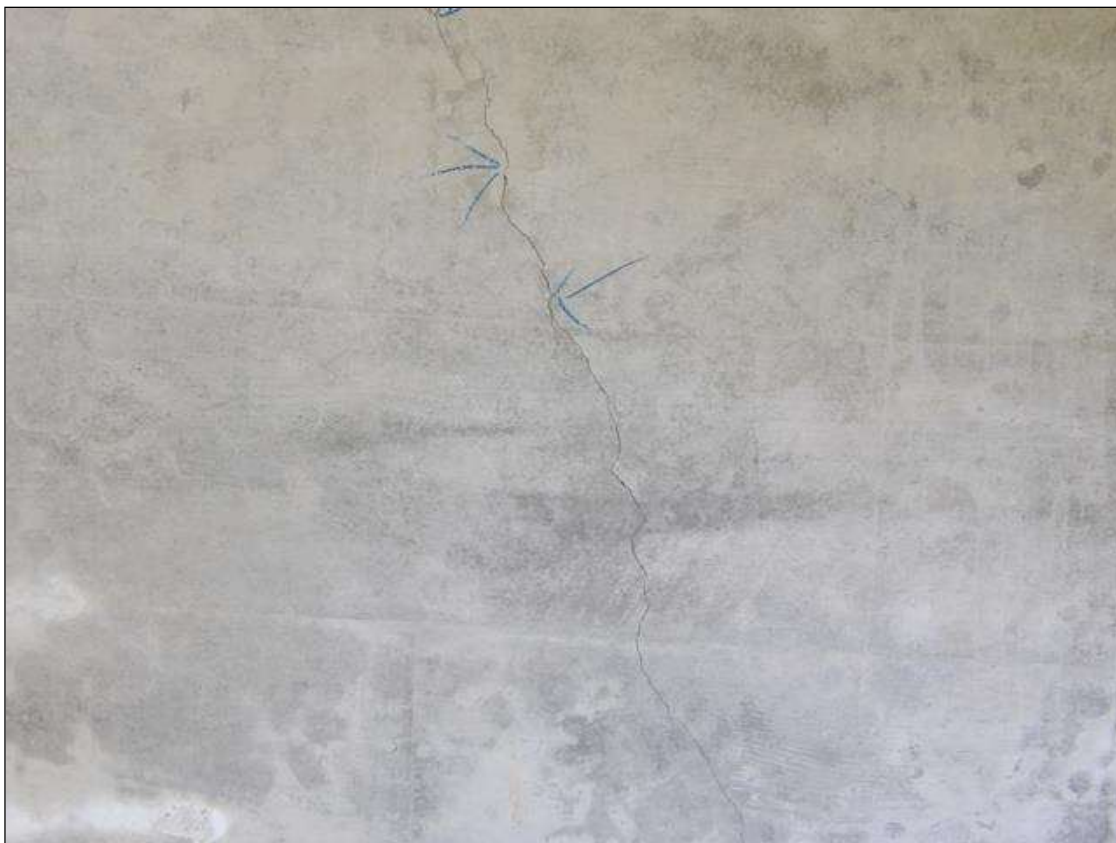
TYPICAL HAIRLINE DIAGONAL CRACKS ON WEB OF BEAM, SPAN 1 BEAM 1 SHOWN
