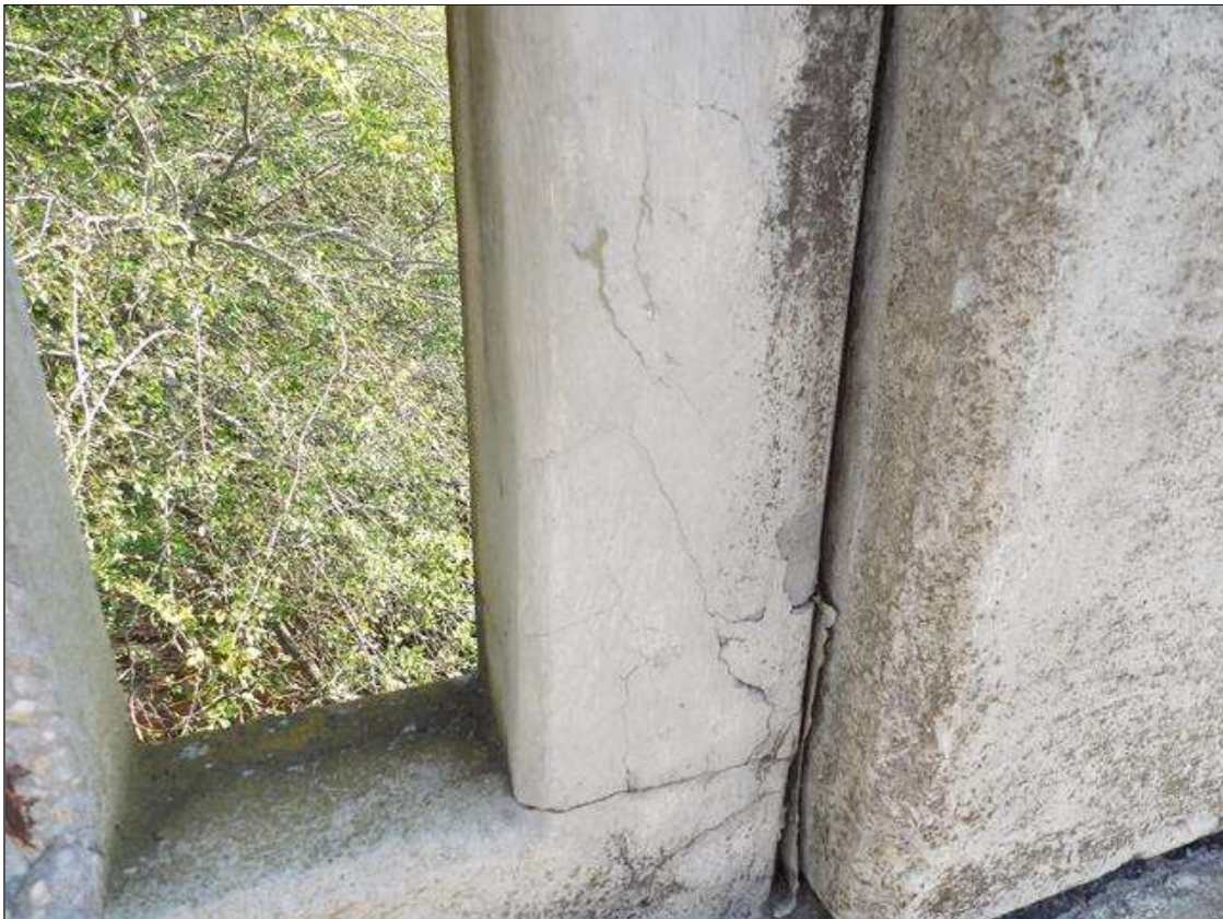
Span 3 Left Bridge Rail: UNSOUND PATCH ON LAST POST OF SPAN 3 LEFT RAIL. FULL FACE OF POST
