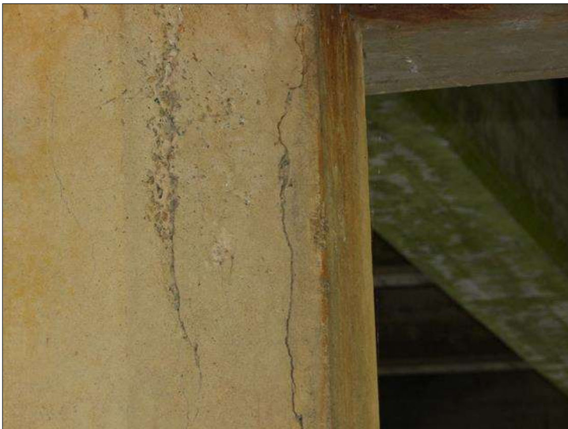
Bent 5 Pile 4: 3' LONG X 4" WIDE AREA OF DELAMINATION EAST FACE AT TOP
