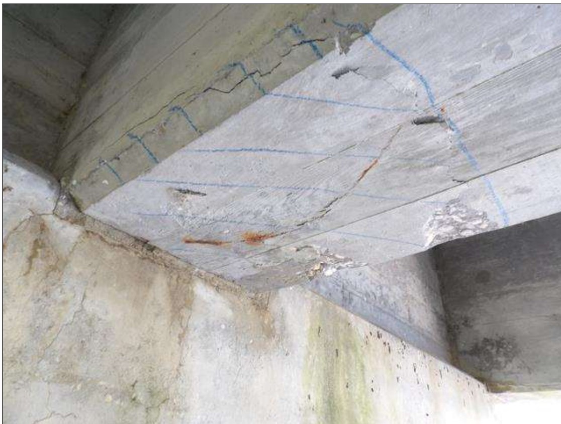
Span 4 Beam 4: 1.5' LONG X FULL WIDTH AREA OF DELAMINATION IN BOTTOM FLANGE AT BENT 4
