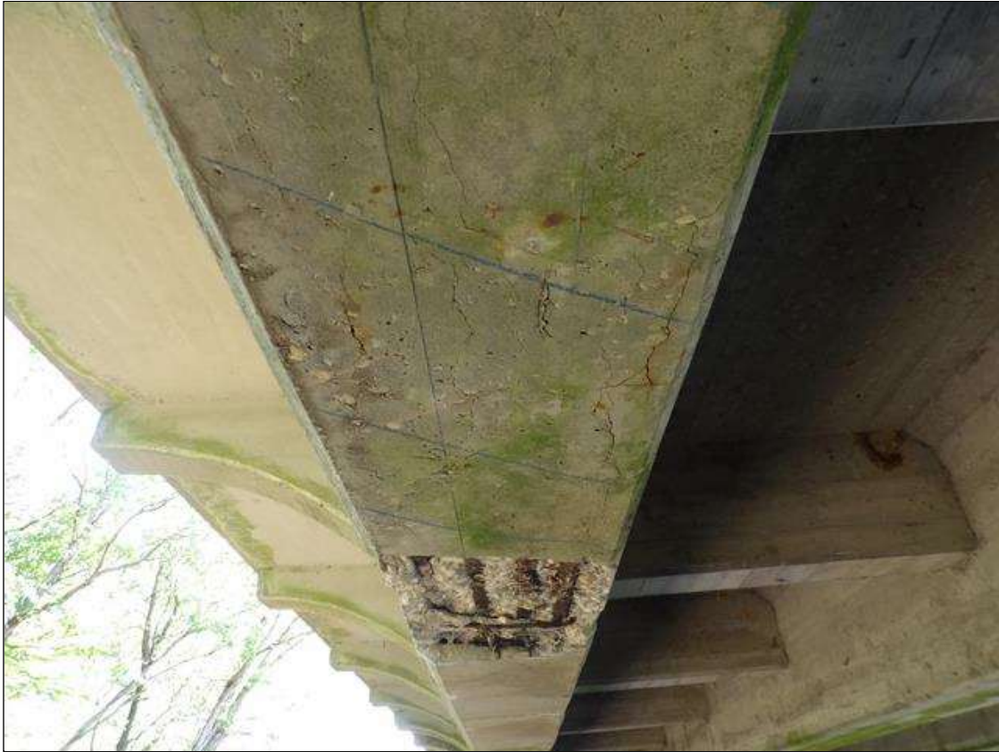
Span 2 Beam 1: PAR -- 12' LONG X FULL WIDTH OF BOTTOM FLANGE EXTENDING 3" ON BOTH FACES AREA OF DELAMINATION WITH 2' LONG X FULL WIDTH X 3" DEEP SPALL WITH EXPOSED REBAR WITH MINIOR SECTION LOSS STARTING 2' FROM BENT 1
