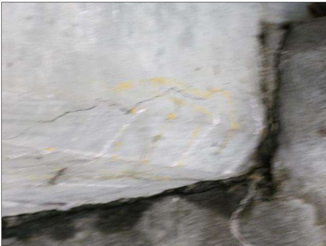
Span 1 Beam 2: AT BENT 1, DELAMINATION 1' LONG X 5" WIDE BOTTOM RIGHT FLANGE
