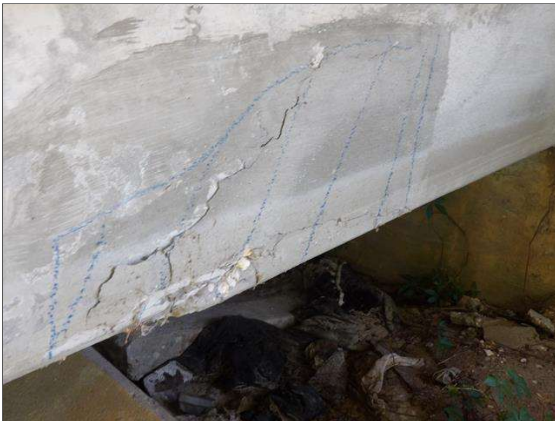
Span 1 Beam 1: 5' FROM END BENT 1, BOTTOM LEFT CORNER DELAMINATION 3' X 2' AREA
