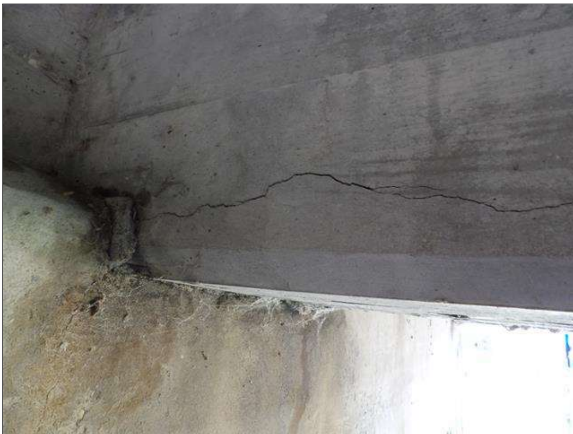
Span 2 Beam 4: 1/8" WIDE X 1' LONG HORIZONTAL CRACK ON BOTTOM LEFT FACE AT BENT 2
