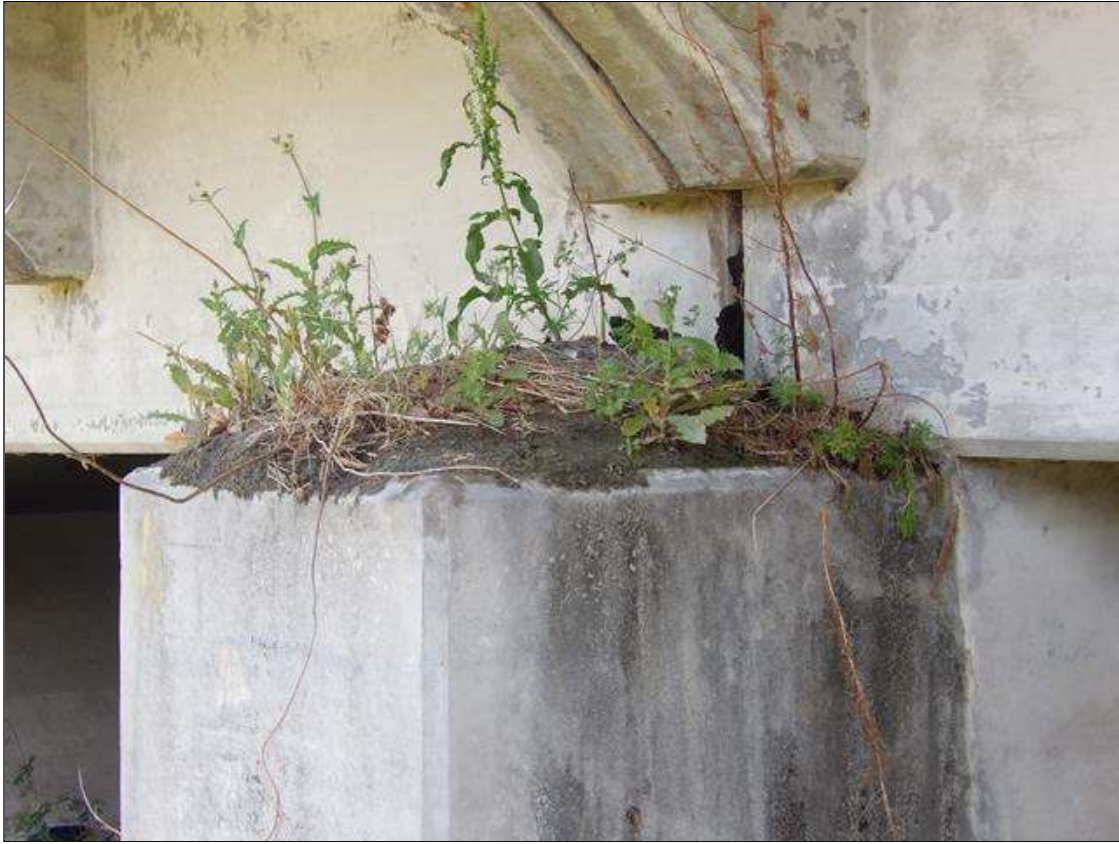
VEGETATION GROWTH ON TOP OF ALL CAPS UNDER OVERHANGS, BENT 1 RIGHT SIDE SHOWN, ALL OTHERS SIMILAR
