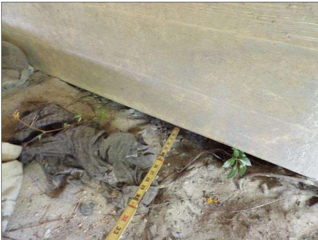
END BENT 1 SLOPE PROTECTION BERM, BELOW BAY 1, CAP 2' WIDE X 6" HIGH X UP TO 21" DEEP VOID CAUSED BY AN ANIMAL
