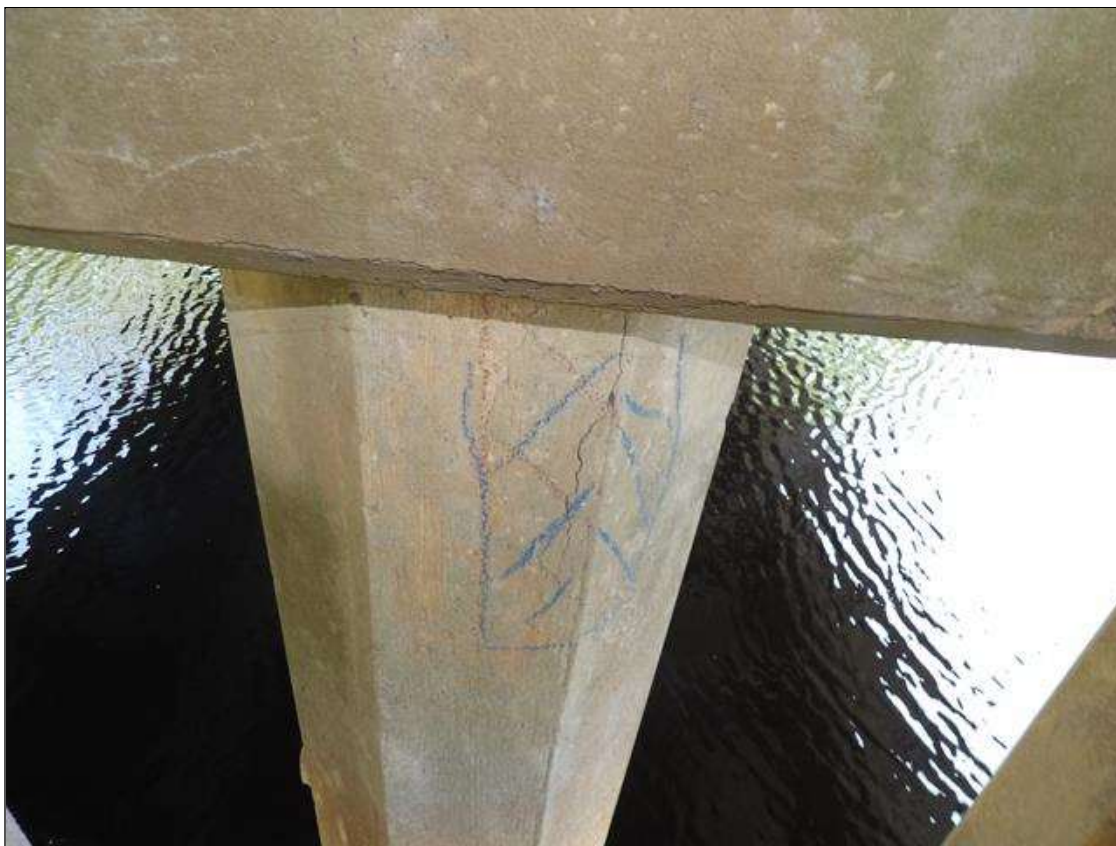
Bent 3 Pile 5: 20" LONG X 16" WIDE AREA OF DELAMINATION ON THE WEST FACE AT TOP OF PILE
