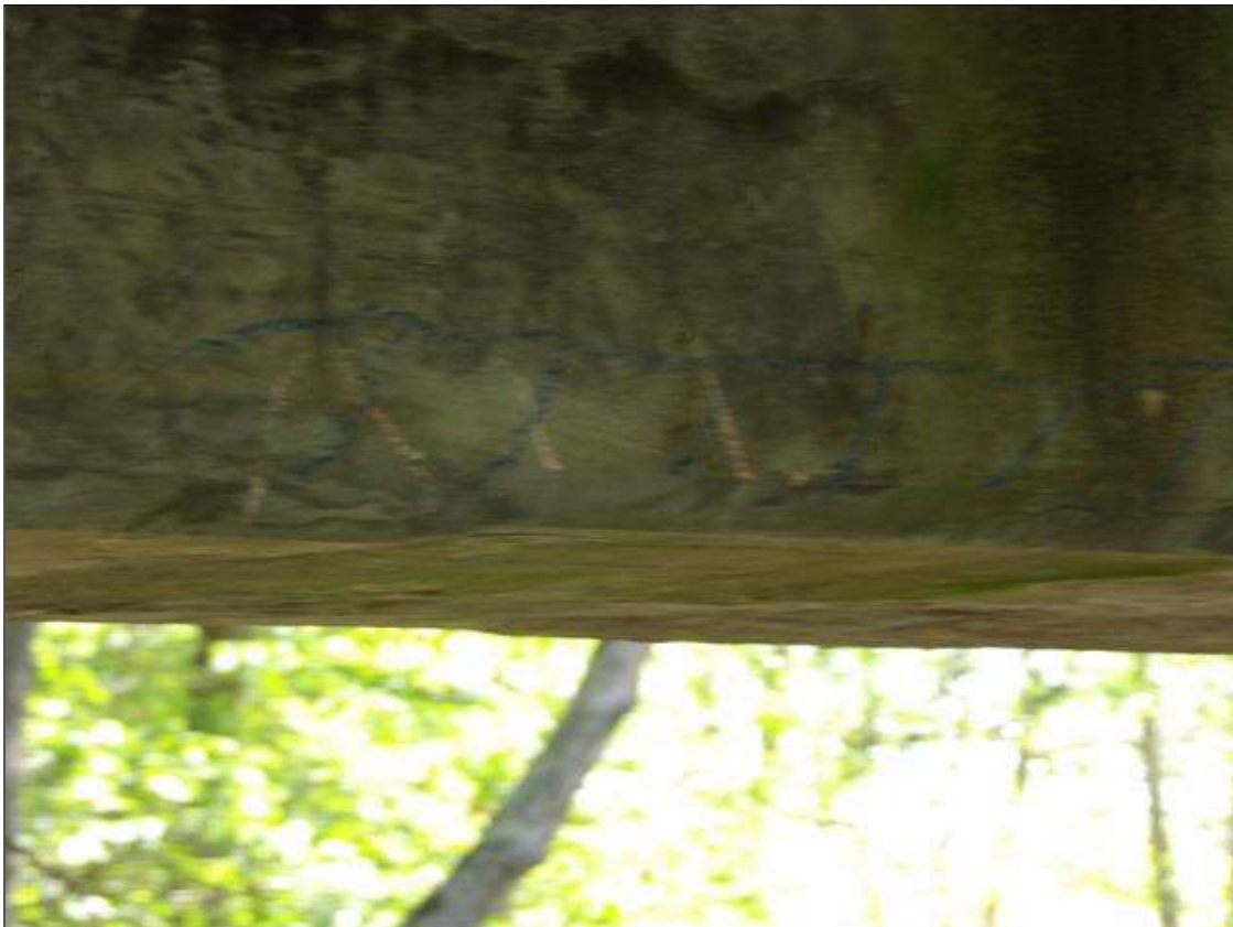
Span 2 Beam 1: 3.5' LONG X 6" WIDE AREA OF DELAMINATION IN BOTTOM RIGHT FACE AT MIDSPAN
