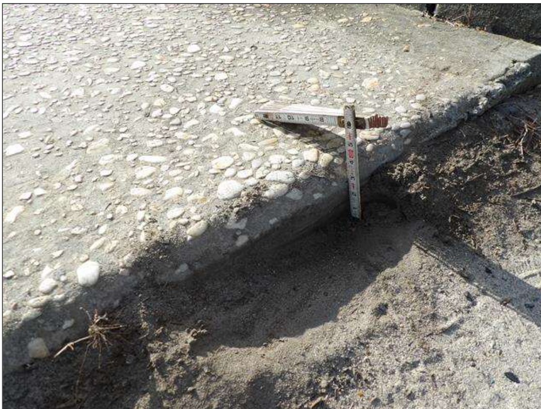
Sidewalk has settled up to 3" x full width at all corners, southwest corner shown
