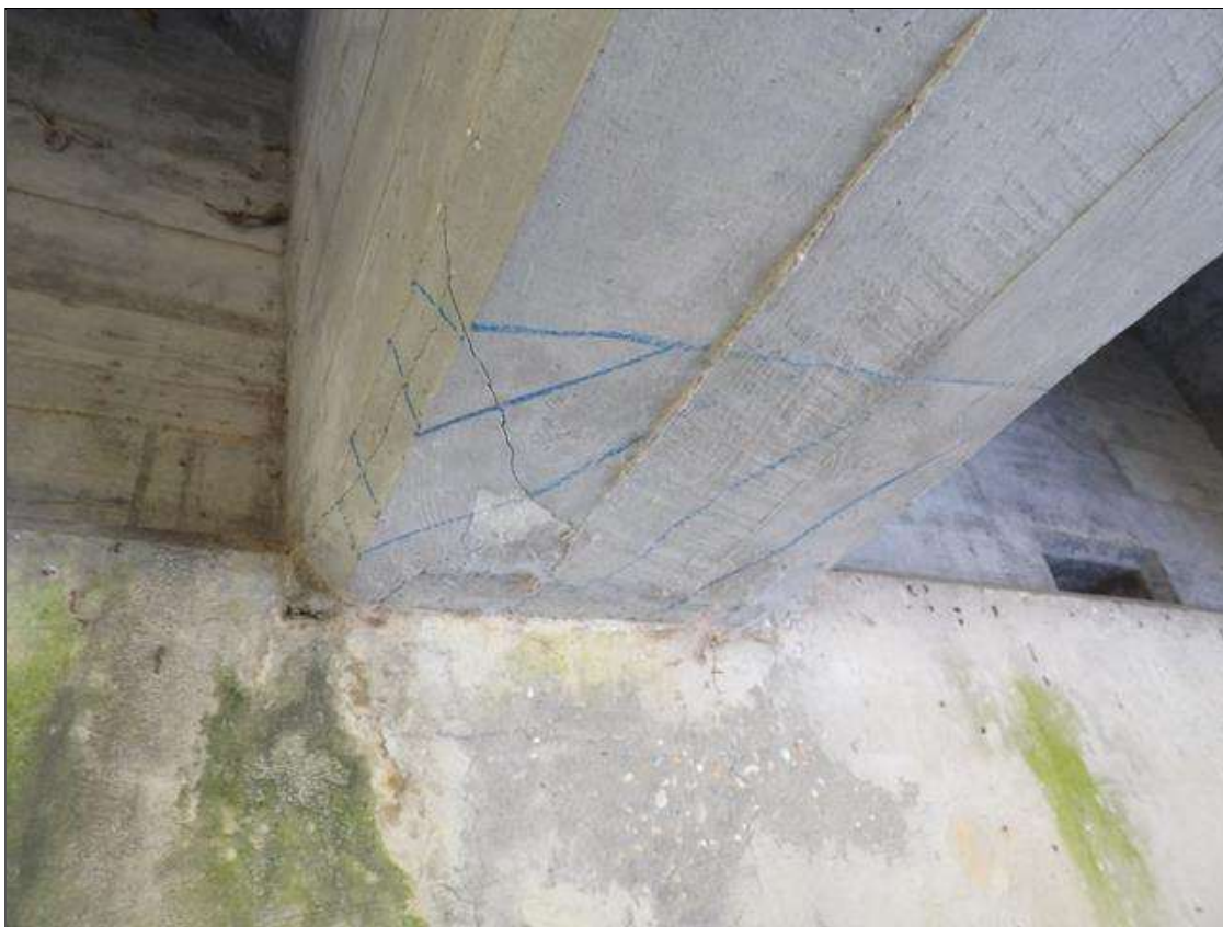
Span 4 Beam 2: 1' LONG X FULL WIDTH AREA OF DELAMINATION IN BOTTOM FLANGE AT BENT 4
