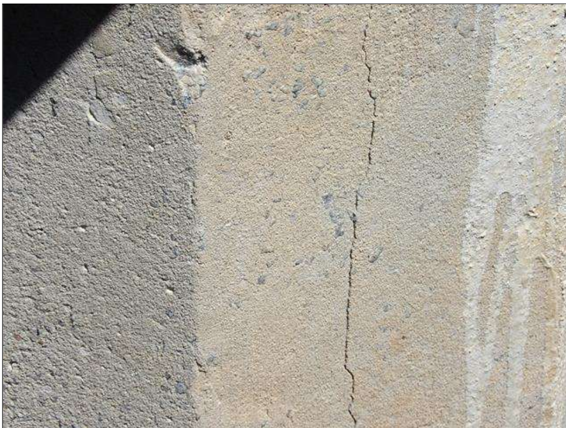
Bent 5 Pile 8: 4' LONG X UP TO 1/16" WIDE VERTICAL CRACK ON SOUTH FACE AT TOP
