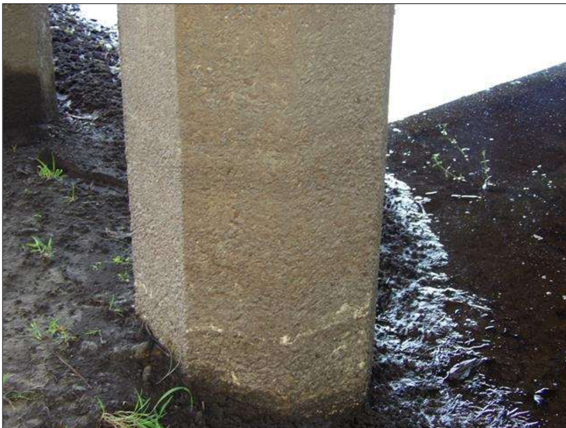
Typical minor abrasion in piles up to 3' high on all faces, Bent 2 Pile 3 shown
