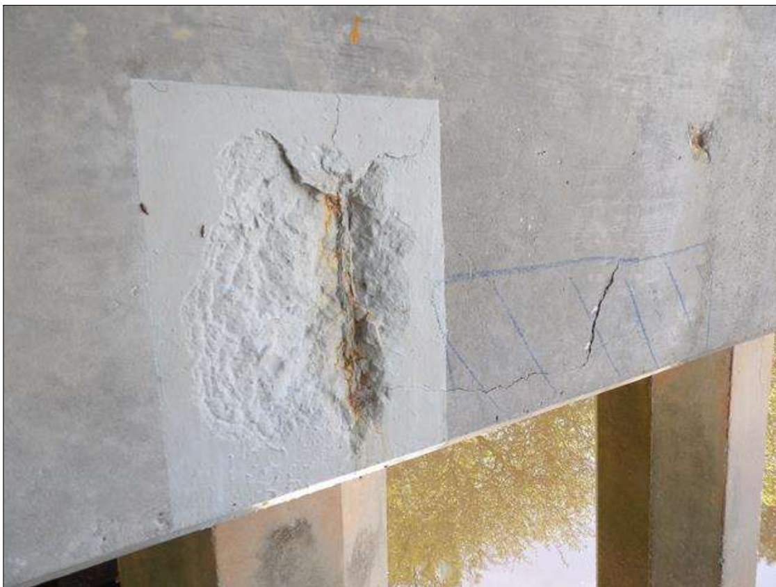
Bent 4 Cap 1: WEST FACE BELOW BEAM 5, 12" HIGH X 18" WIDE X 2" DEEP SPALL WITH EXPOSED REBAR. AREA HAS BEEN COATED AND STEEL IS NOT CORRODED. ADJACENT 24" X 16" DELAMINATION
