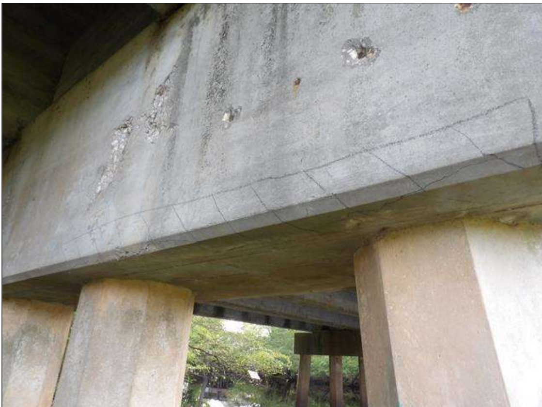
Bent 2 Cap 1: DELAMINATION ON NEAR FACE AT BOTTOM OF CAP 4' LONG X 6" HIGH.
