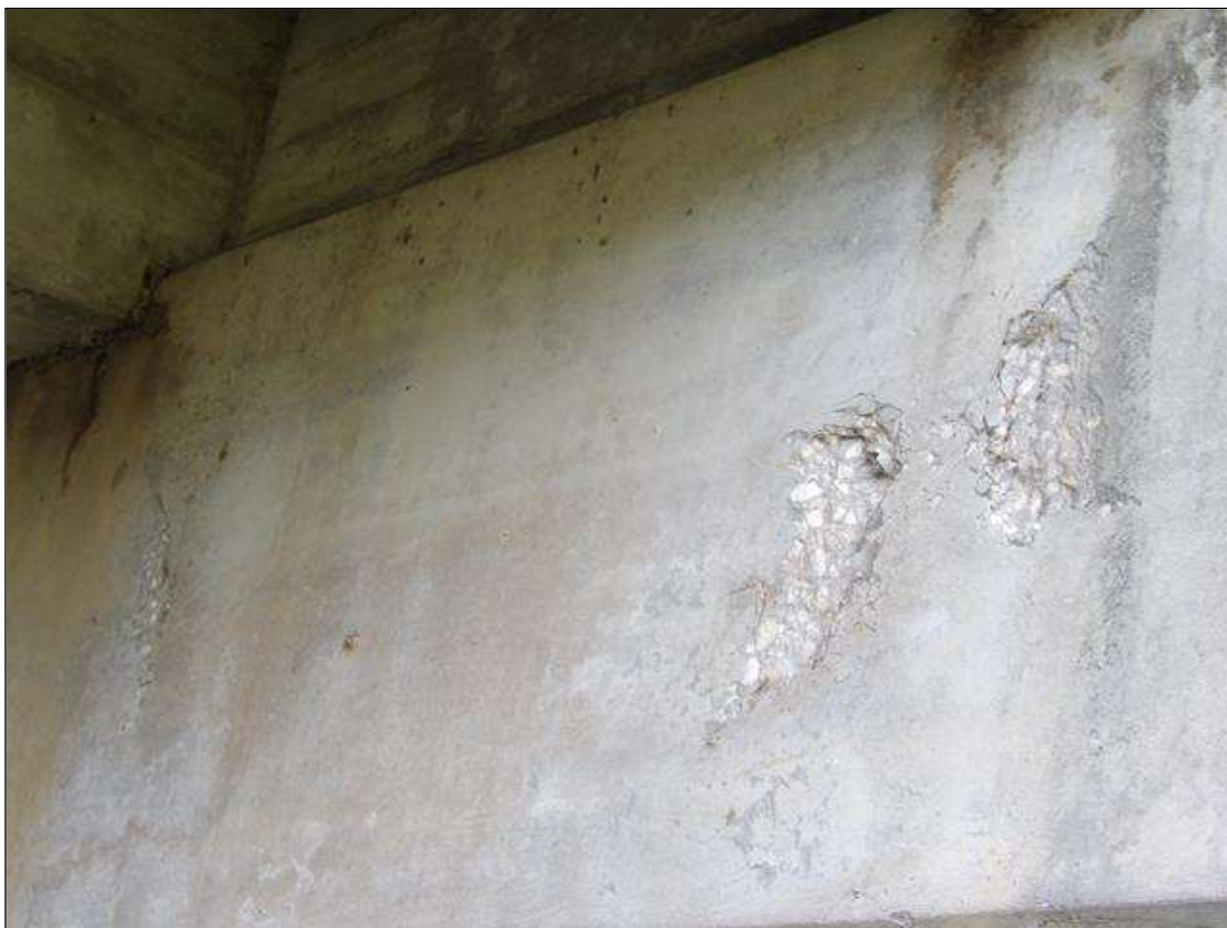
Bent 2 Cap 1: NEAR FACE, (6) SPALLS UP TO 12" LONG X 4" WIDE X 1" DEEP UNDER BEAMS 4 AND 5.
