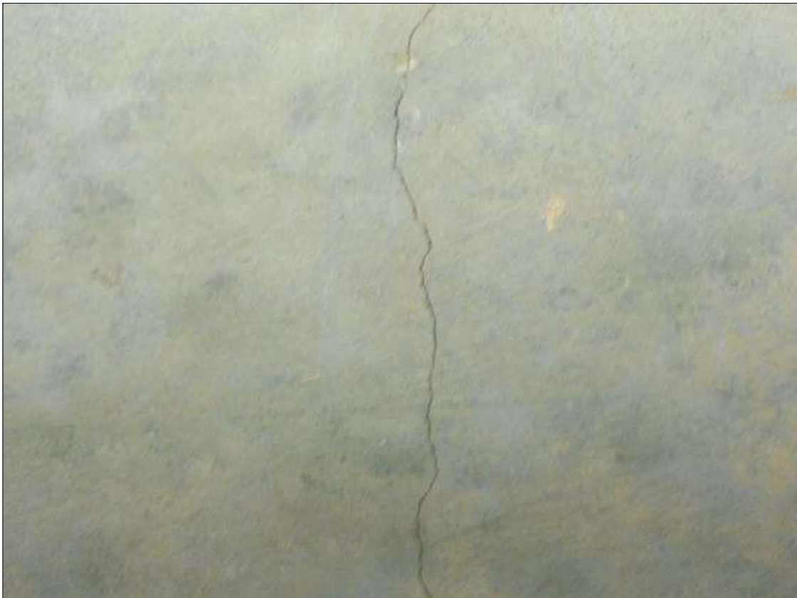
End Bent 1 Cap 1: 2 FULL HEIGHT X HAIRLINE TO 1/32" WIDE VERTICAL CRACKS AT BAY 2 AND 3
