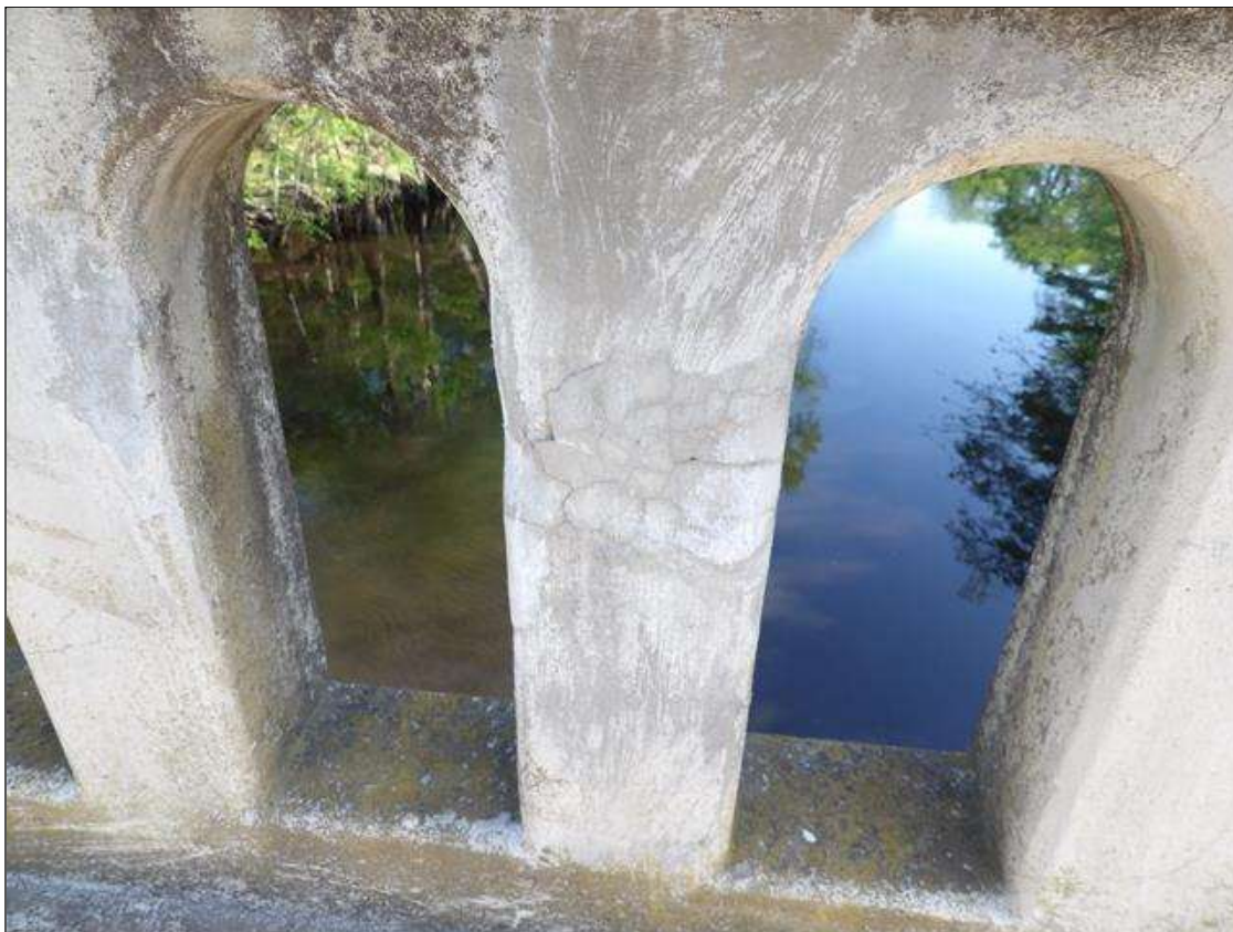
Span 5 Left Bridge Rail: 4TH POST FROM BENT 5 UNSOUND PATCH ON TOP HALF OF INTERIOR FACE. PATCH IS DELAMINATED.
