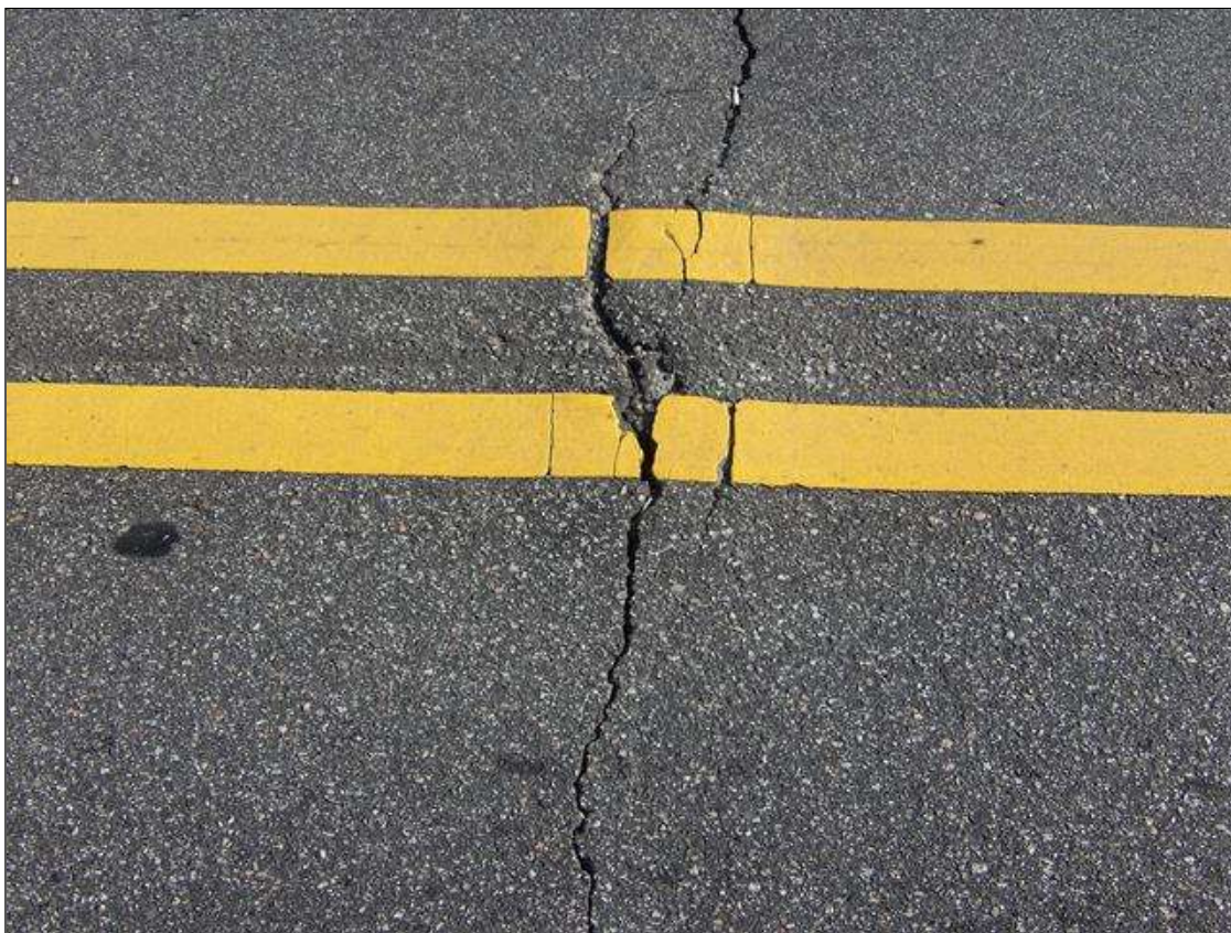
TYPICAL TRANSVERSE CRACKS UP TO FULL WIDTH X 1/2" WIDE, OVER BENT 3 SHOWN
