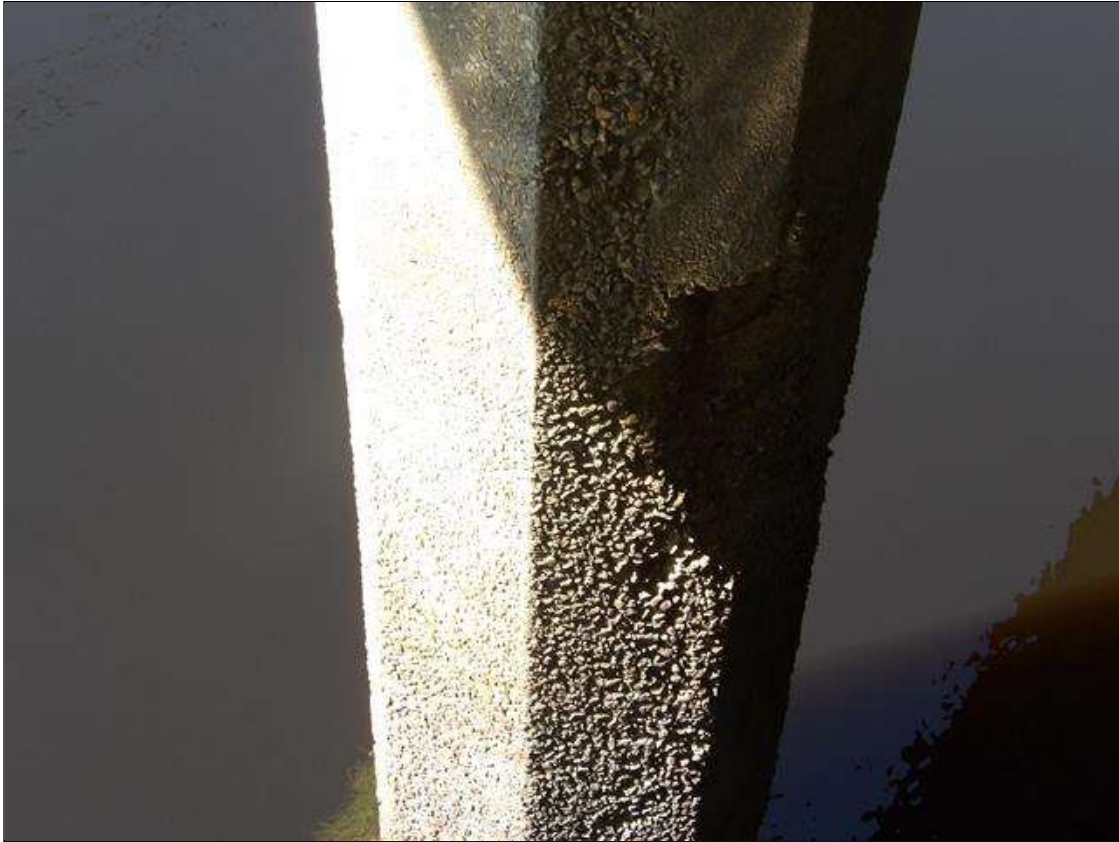
Bent 3 Pile 8: 5' BELOW THE CAP, 3' LONG X 12" WIDE X 2" DEEP WITH EXPOSED REBAR WITH NO MEASURABLE SECTION LOSS
