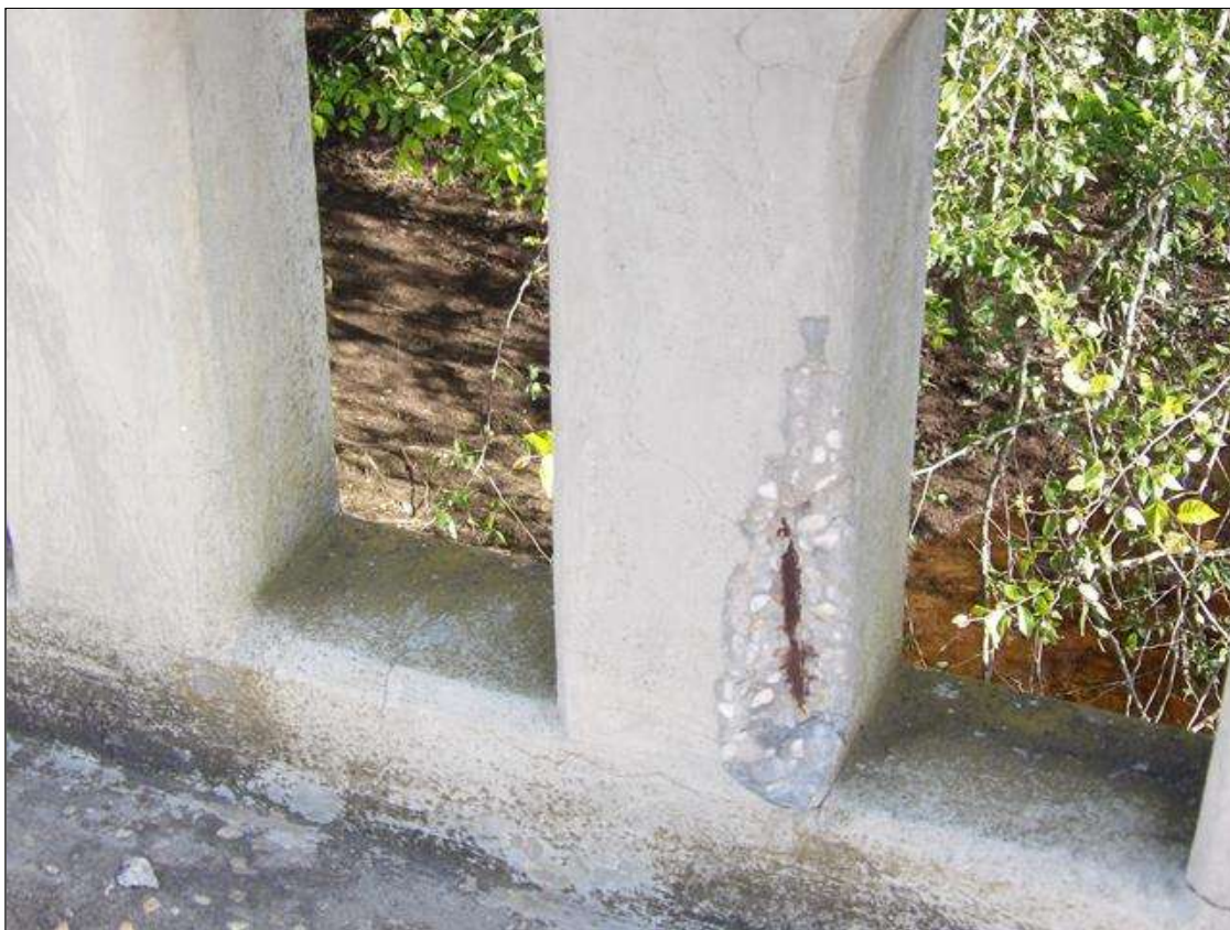
Span 3 Left Bridge Rail: SPALL ON 2ND POST FROM BENT 3, SOUTH FACE, 3" LONG X 12" HIGH X 2" DEEP WITH EXPOSED REBAR WITH NO SECTION LOSS
