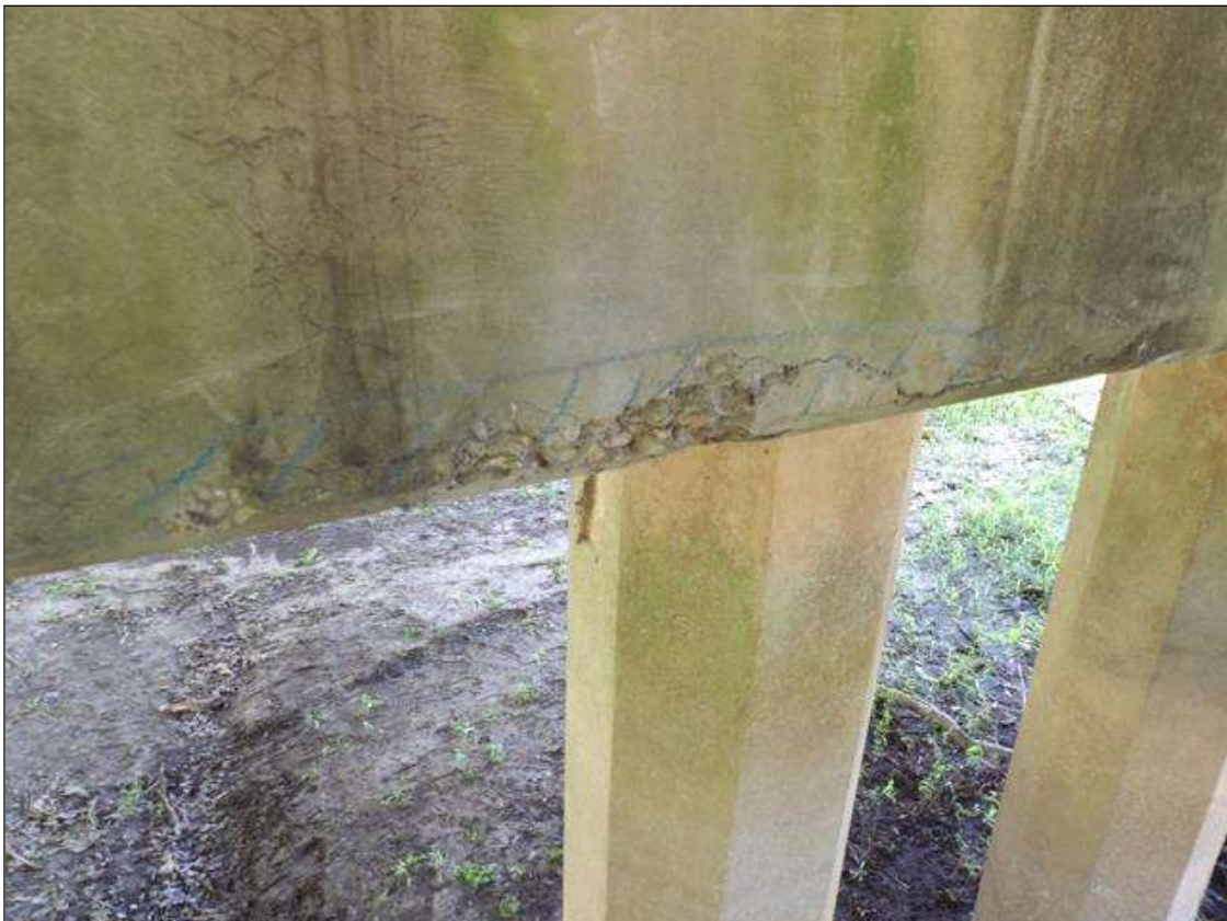
Bent 2 Cap 1: 2' LONG X 4" HIGH DELAMINATION WITH DETERIORATED CONCRETE AND CRACKS UNDER BEAM 2
