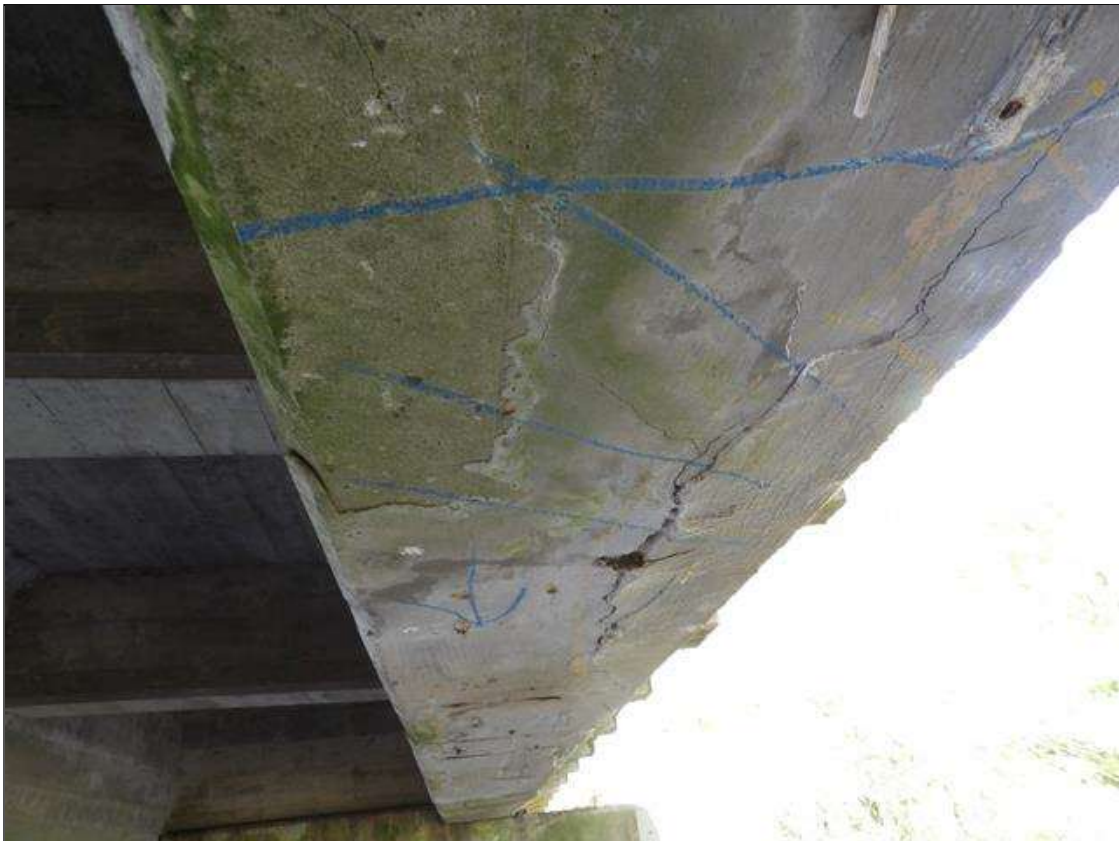
Span 5 Beam 1: 20' LONG X FULL WIDTH AREA OF DELAMINATION IN BOTTOM FLANGE EXTENDING UP TO 2' IN BOTH FACES OF WEB, STARTING 3' FROM BENT 4
