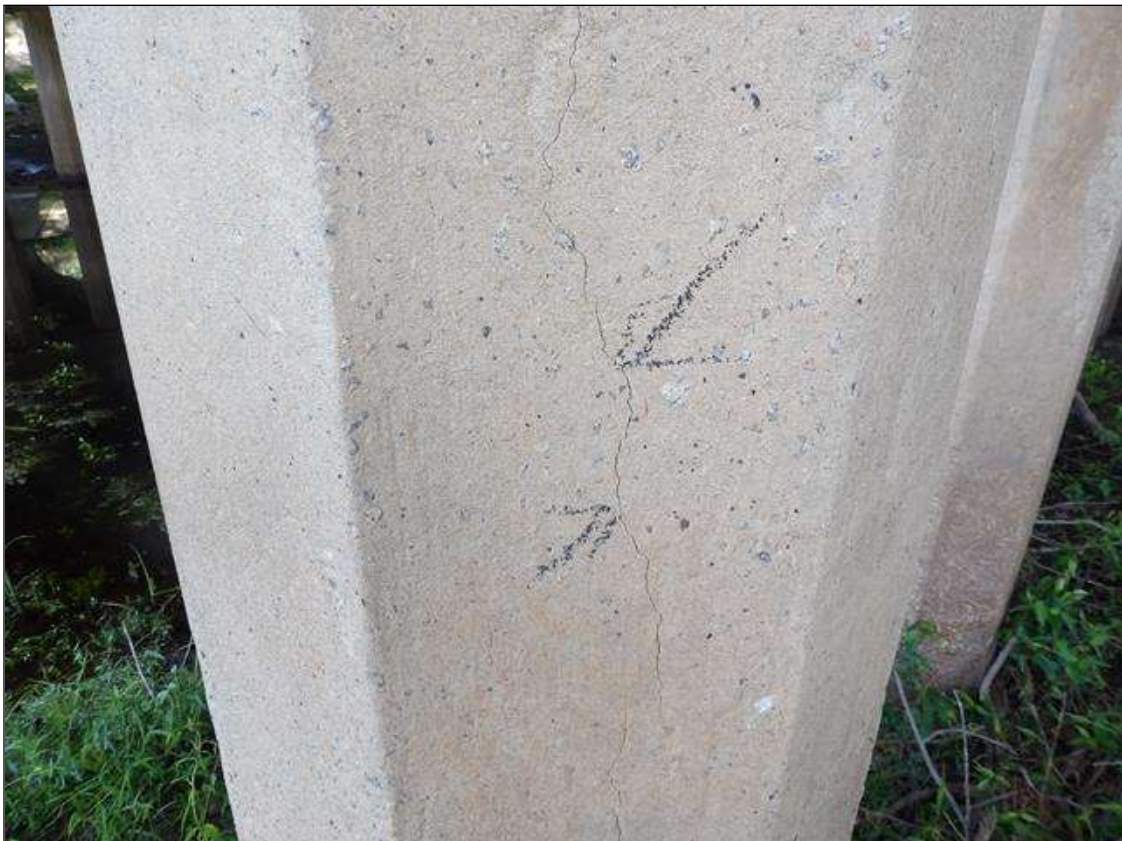
Typical vertical hairline crack on Piles, Bent 2 Pile 7 shown
