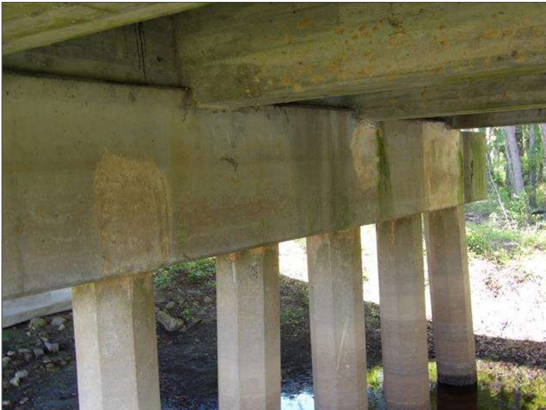
Bent 1 Cap 1: (3) SOUND PATCHS UP TO 4' LONG X 3' WIDE ON EAST FACE AT VARIOUS LOCATIONS
