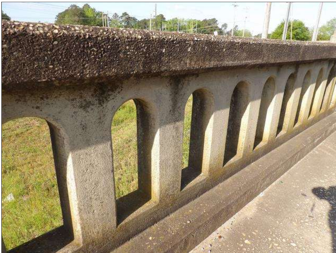
Typical sound patch interior face of rail post, Span 1 right rail shown
