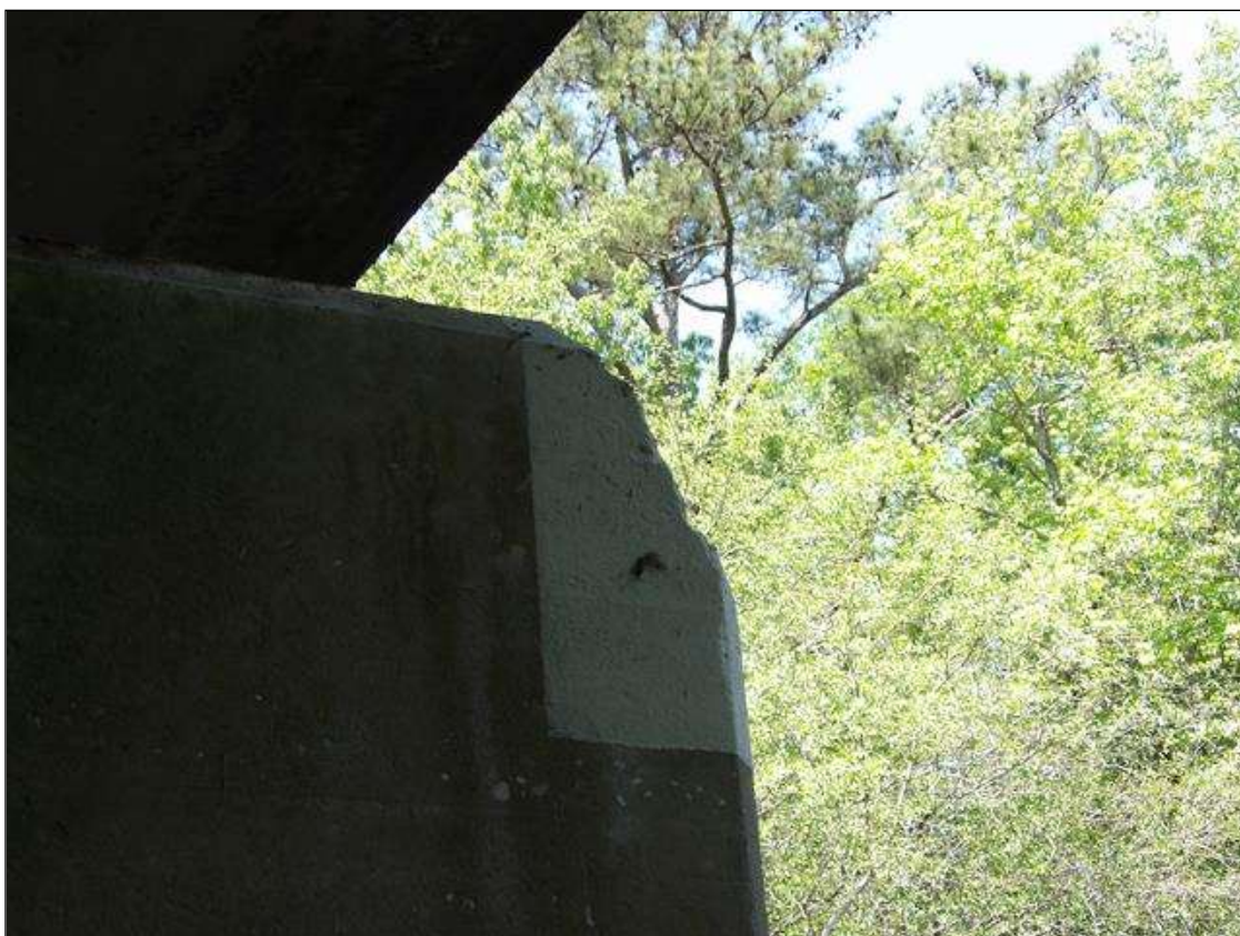
Bent 4 Cap 1: CORNER SPALL ON LEFT END TOP, 1' LONG X 10" WIDE X 3" DEEP, PREVIOUSLY COATED AREA
