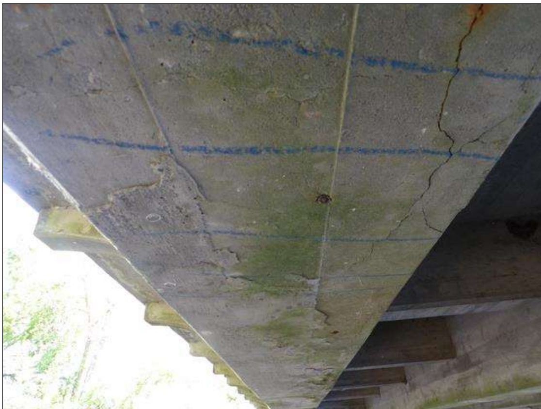
Span 4 Beam 1: 25' LONG X FULL WIDTH AND EXTENDING UP TO 3" HIGH ON BOTH FACES AREA OF DELAMINATION STARTING 5' FROM BENT 3
