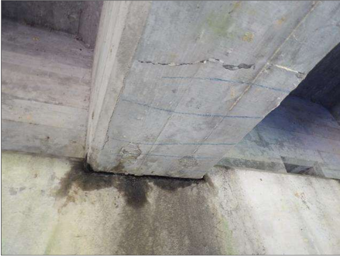
Span 2 Beam 2: 2' LONG X FULL WIDTH AREA OF DELAMINATION IN BOTTOM FACE AT BENT 2
