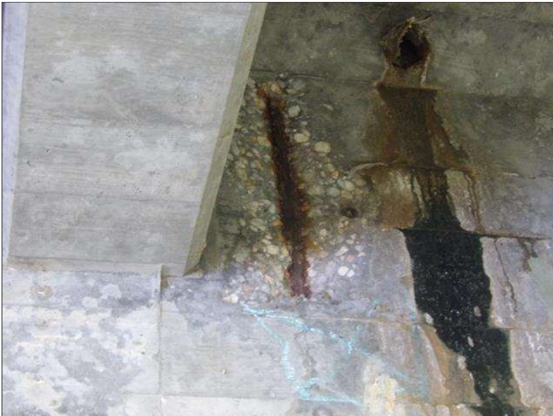
Span 6 Beam 1: PAR -- 20" LONG X 12" WIDE X 1" DEEP SPALL WITH EXPOSED REBAR WITH MINOR SECTION LOSS AND 10" DIA. AREA OF DELAMINATION BELOW SPALL, IN RIGHT FACE AT DIAPHRAGM
