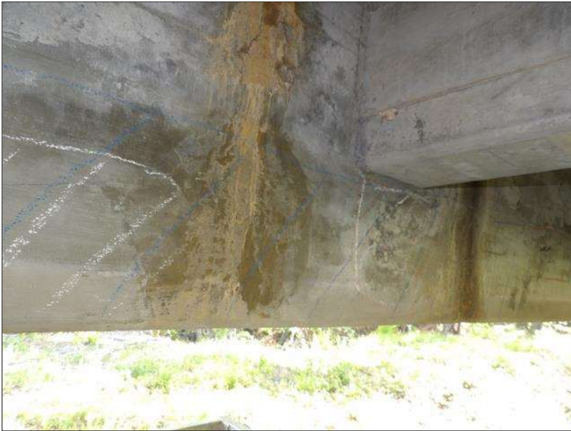
Span 1 Beam 1: 12' LONG X UP TO 2' WIDE AREA OF DELAMINATION IN RIGHT FACE NEAR MIDSPAN
