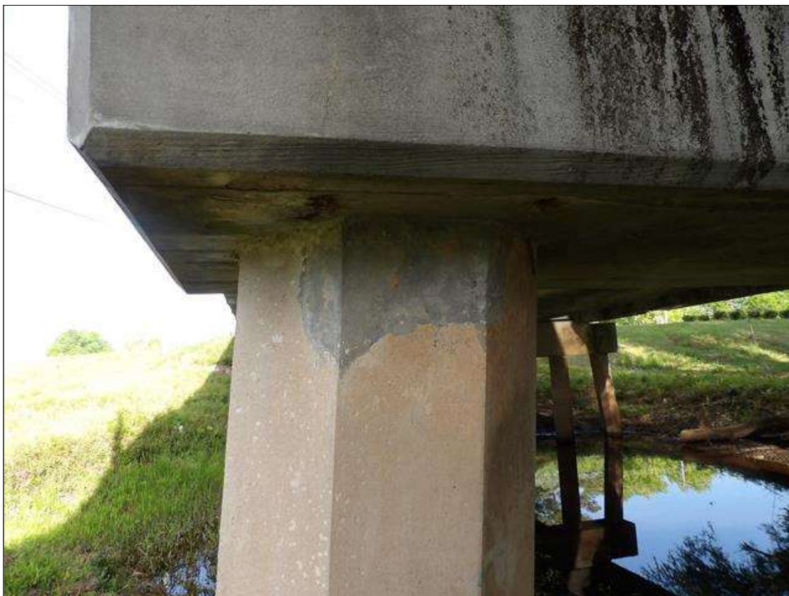
Bent 2 Pile 8: 1' x 8" SOUND PATCH AT TOP OF PILE ON EAST FACE
