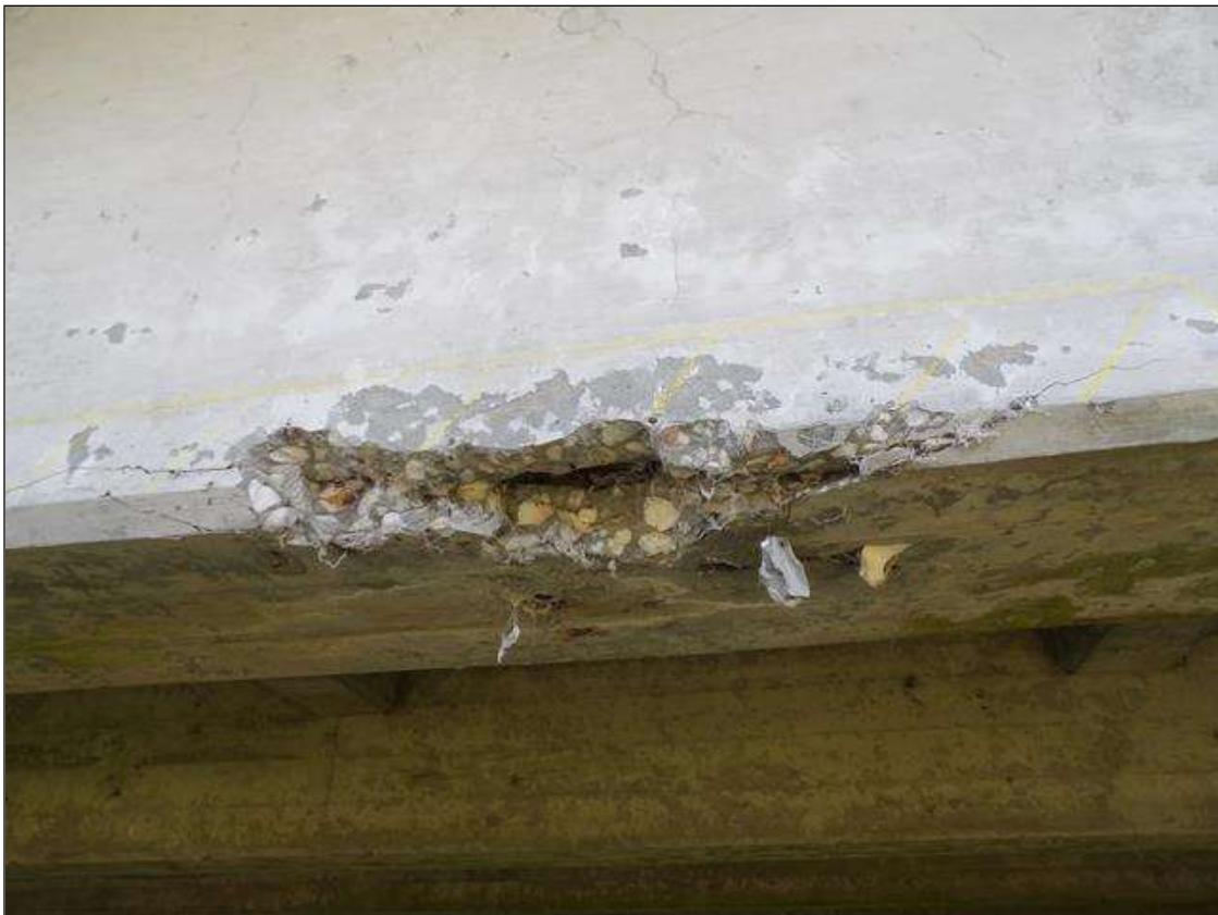
Span 1 Beam 5: PAR - 9' FROM BENT 1, BOTTOM OF BEAM BOTH SIDES, SPALL AND DELAMINATION 5' LONG X 6" HIGH X 3" DEEP WITH EXPOSED REBAR WITH MINOR SECTION LOSS
