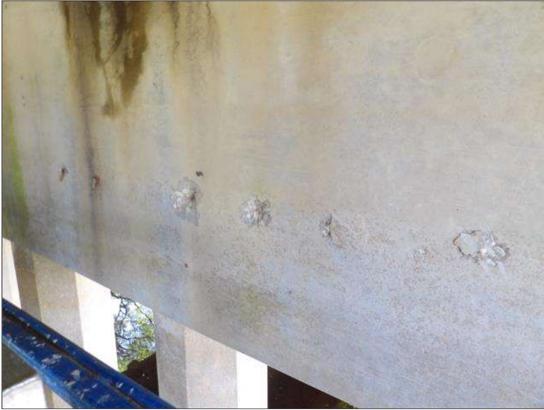
Bent 1 Cap 1: (15) UP TO 5" DIAMETER X 1" DEEP ROUND POP OUT SPALLS WITH EXPOSED REBAR WITH NO MEASURABLE SECTION LOSS ON WEST FACE
