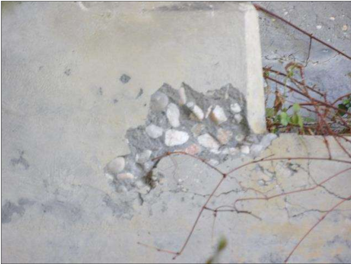
End Bent 2 Cap 1: 3" HIGH X 4" LONG X 1" DEEP SPALL, NO EXPOSED REBAR AT BEAM 5
