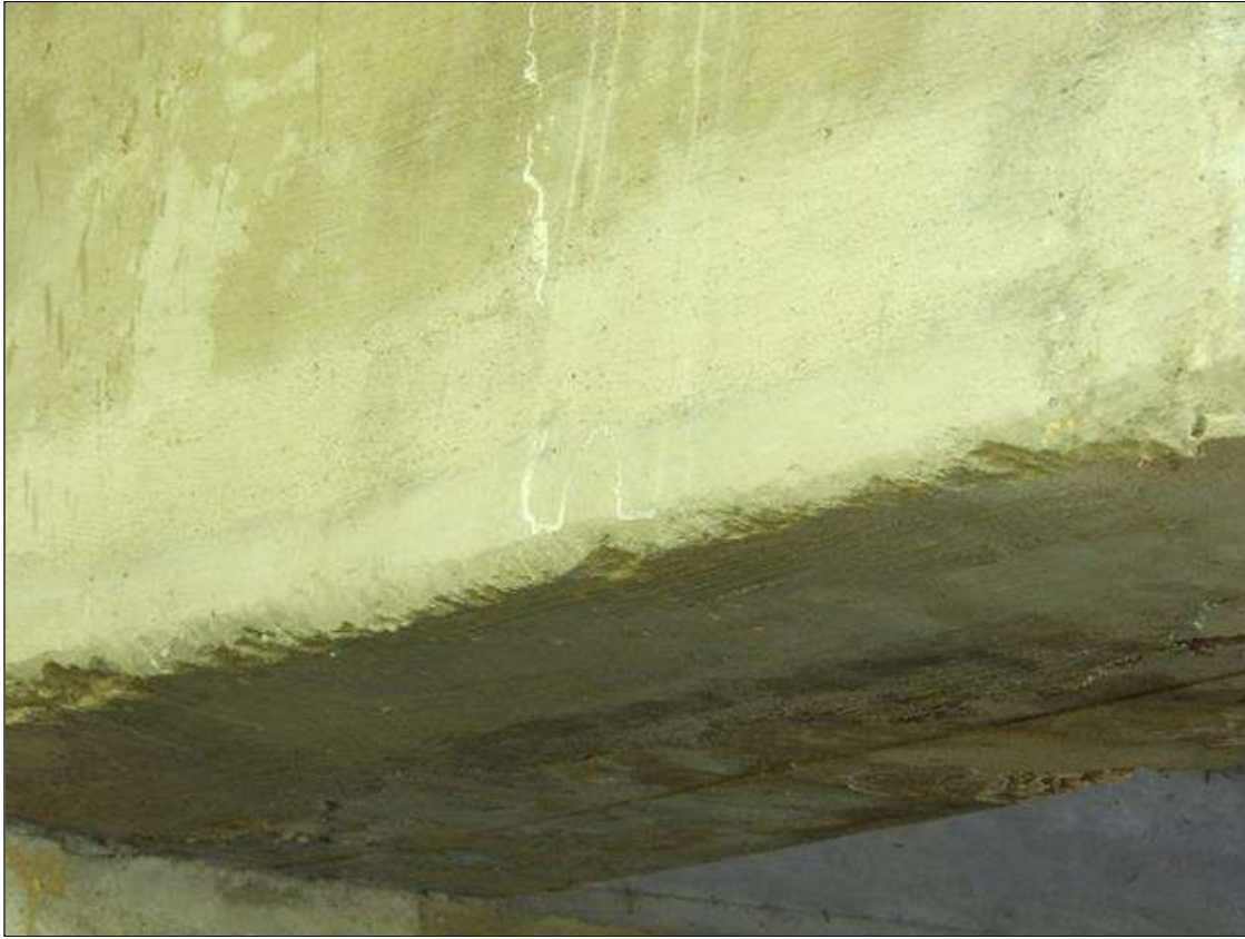
Span 6 Beam 1: 4' LONG X 5" SOUND PATCH ON LEFT FACE OF BEAM LOCATED 5' FROM END BENT 2
