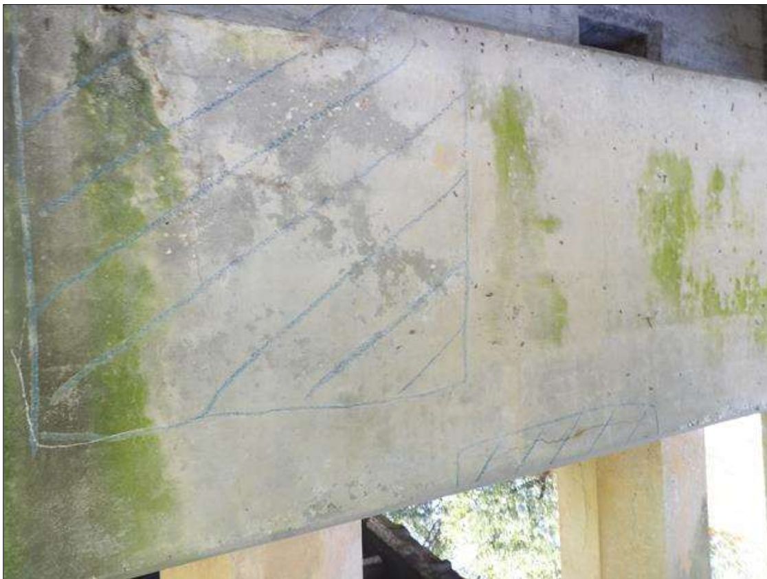
Bent 4 Cap 1: (2) AREAS OF DELAMINATION IN WEST FACE OF CAP IN BAY 2, UP TO 3' LONG X 3' WIDE
