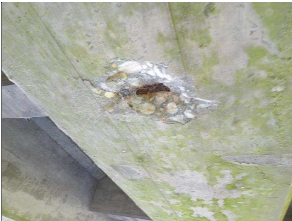
Span 5 Beam 2: (2) 5" DIA. X 1" DEEP SPALLS WITH EXPOSED REBAR IN BOTTOM FLANGE AT 5' AND 10' FROM PIER 5
