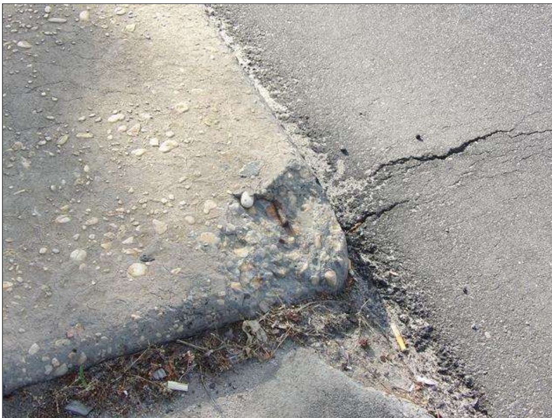
Span 1 Left Bridge Rail: 10" long x 7" wide x 2" deep with exposed rebar with no measurable section loss in sidewalk at abutment 1
