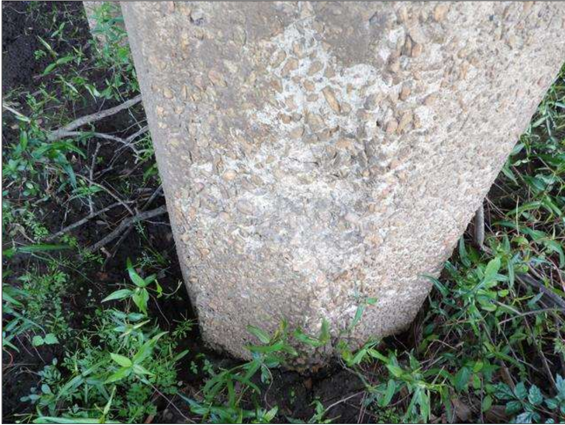
Bent 2 Pile 6: AREA OF DELAMINATION CONCRETE. 8"DIAMETER X 1"DEEP.
