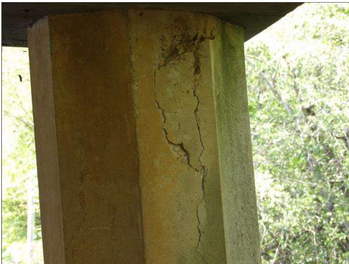
Bent 5 Pile 1: 3' LONG X 4" WIDE AREA OF DELAMINATION EAST FACE AT TOP
