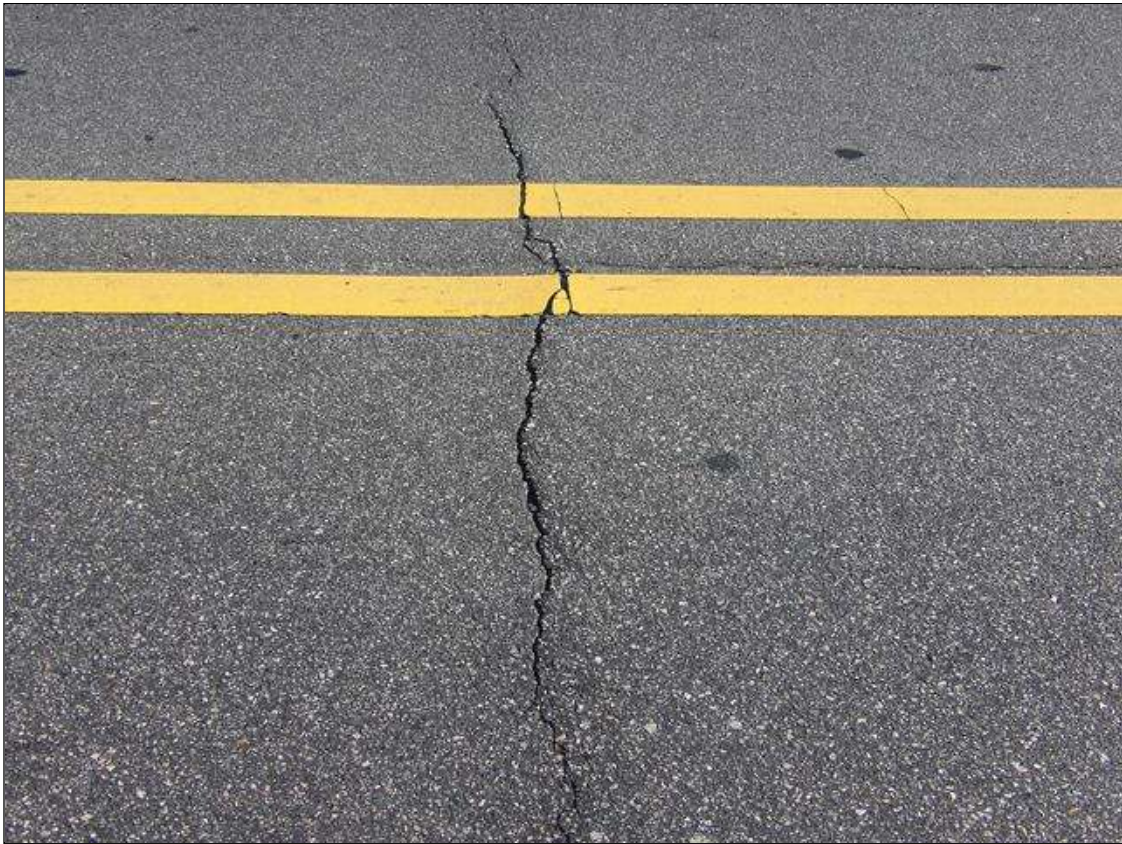
TYPICAL TRANSVERSE CRACK IN WEARING SURFACE FULL LENGTH X UP TO 1/4" WIDE, OVER ABUTMENT 1 SHOWN
