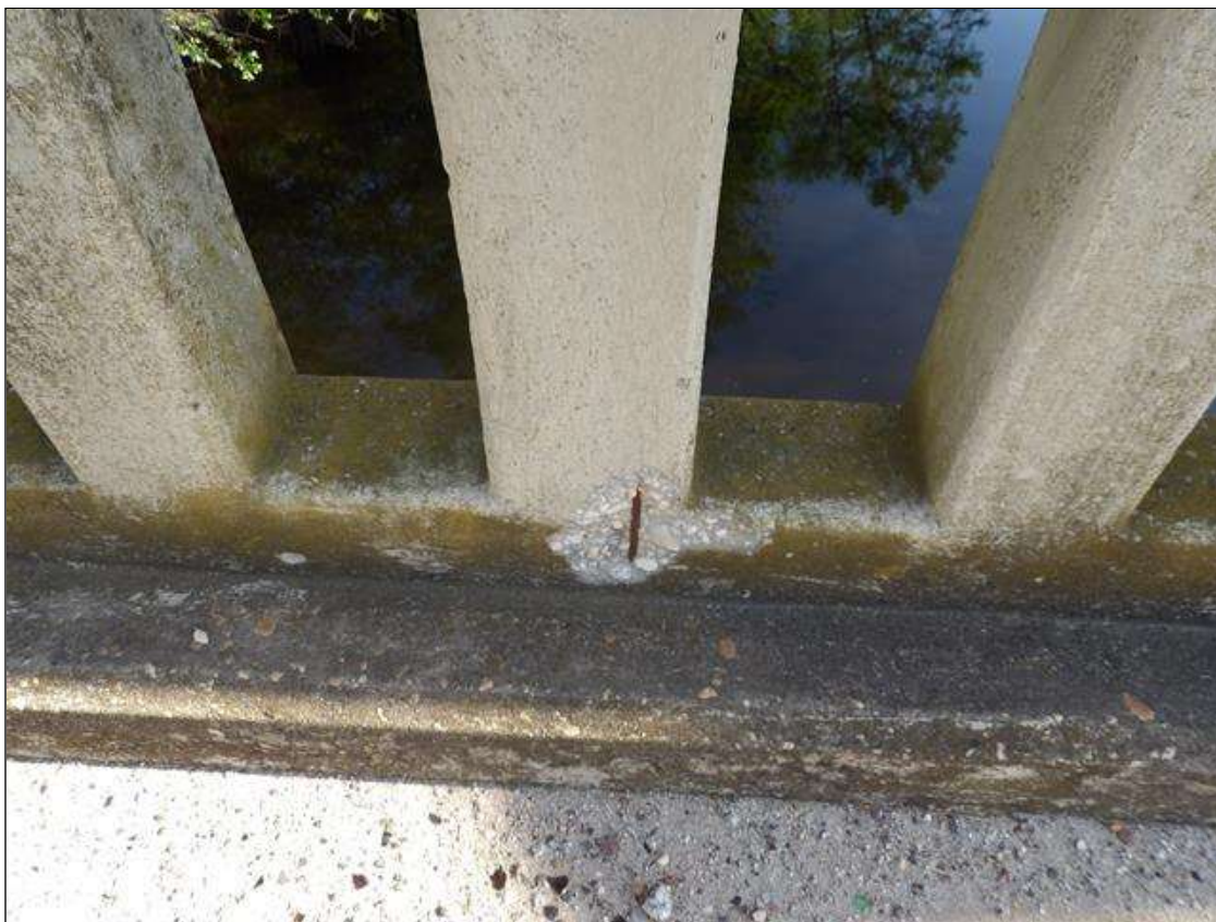
Span 4 Left Bridge Rail: 6" DIAMETER X 1" DEEP SPALL WITH EXPOSED REBAR WITH NO SECTION LOSS. LOCATED AT MIDSPAN LEFT RAIL SPAN 4
