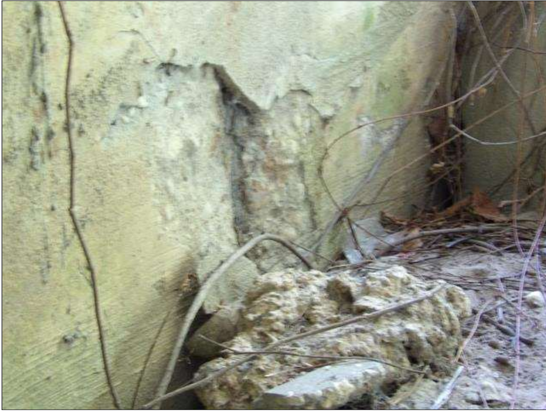
End Bent 1 Cap 1: PAR -- SPALL 16" X UP TO 12" X UP TO 1" DEEP UNDER LEFT OVERHANG WITH EXPOSED REBAR 5" LONG
