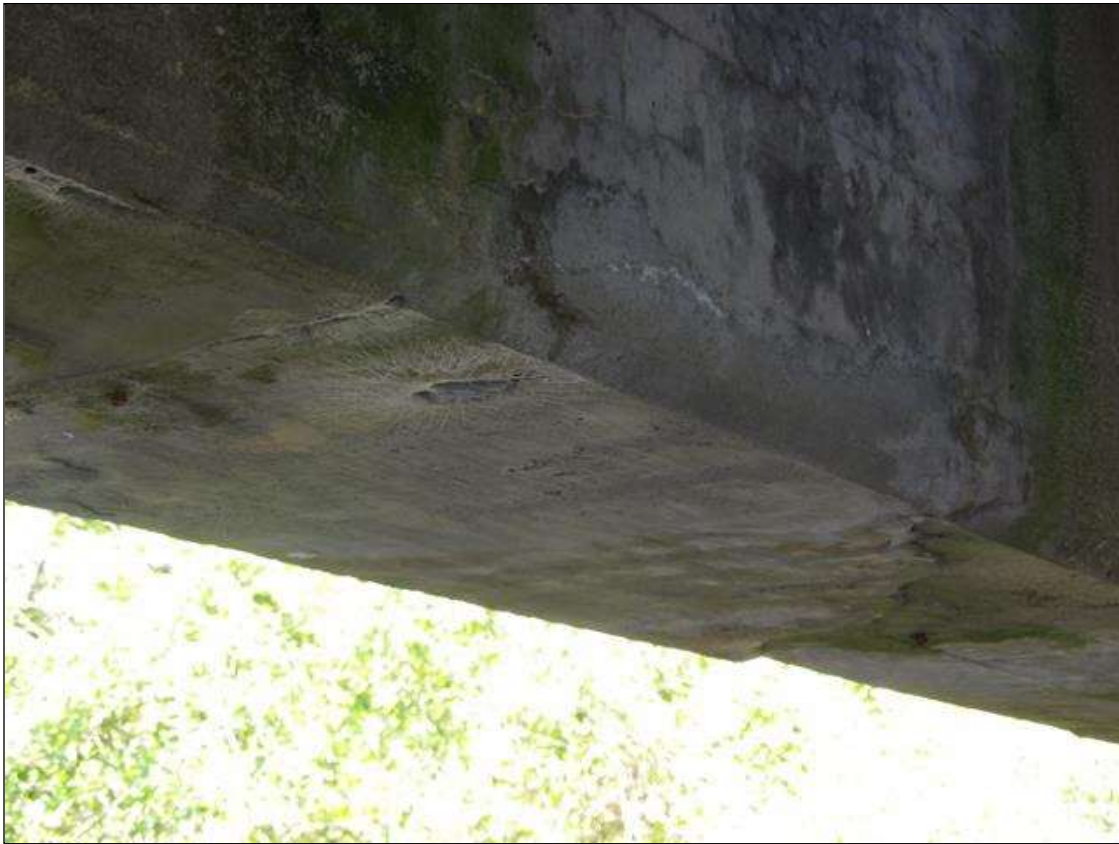
Span 5 Beam 1: SOUND PATCH 24" LONG X 10" HIGH ON RIGHT FACE IN THE WEB AREA NEAR MID SPAN
