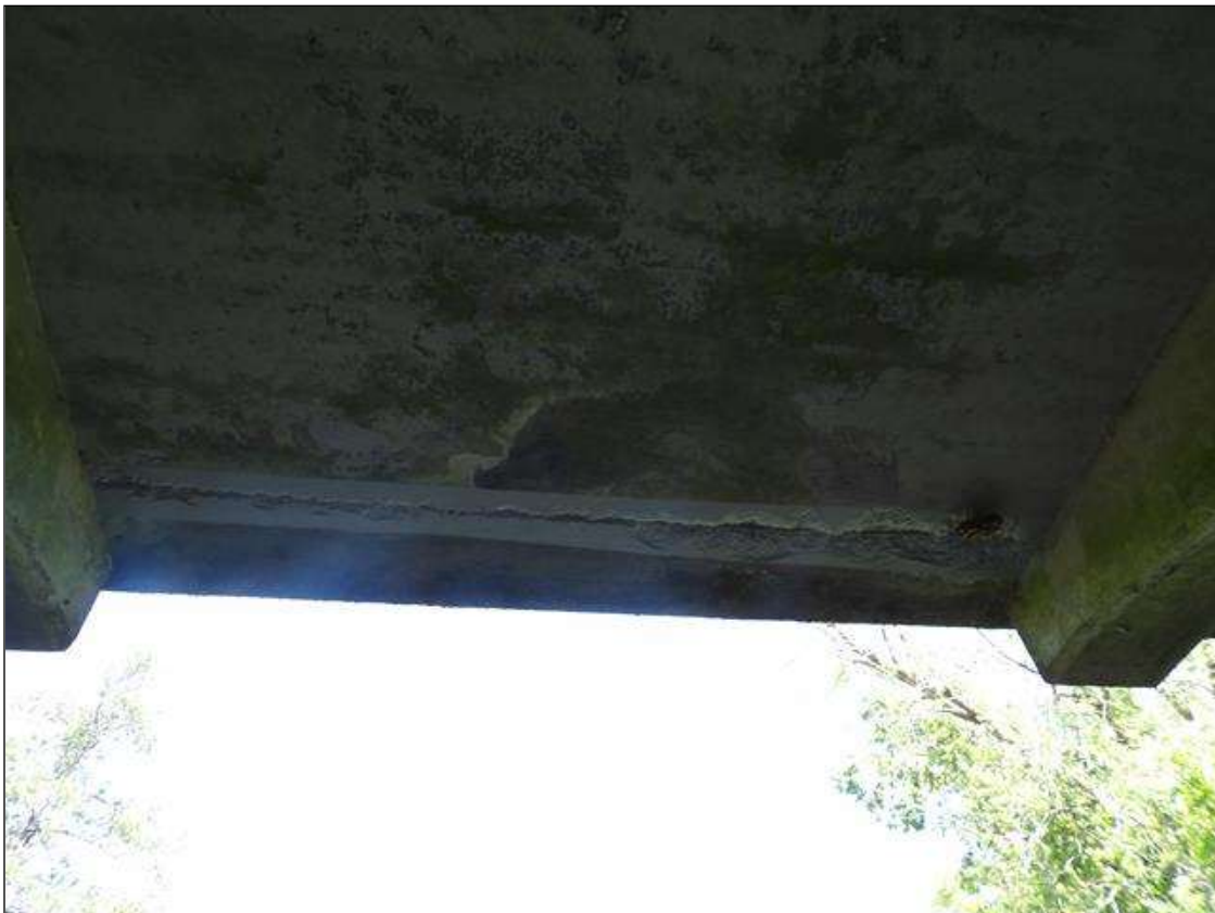
Span 5 Deck: 6' LONG X 7" WIDE X 1" DEEP SPALL WITH EXPOSED REBAR IN DECK UNDERSIDE LEFT OVERHANG. AREA HAS BEEN PAINTED OVER
