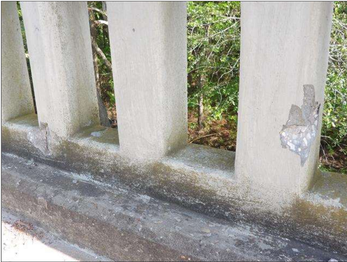
Span 3 Left Bridge Rail: (2) SPALLS UP TO 6" DIA. X 2" DEEP WITH EXPOSED REBAR WITH NO MEASURABLE SECTION LOSS IN RAIL POSTS
