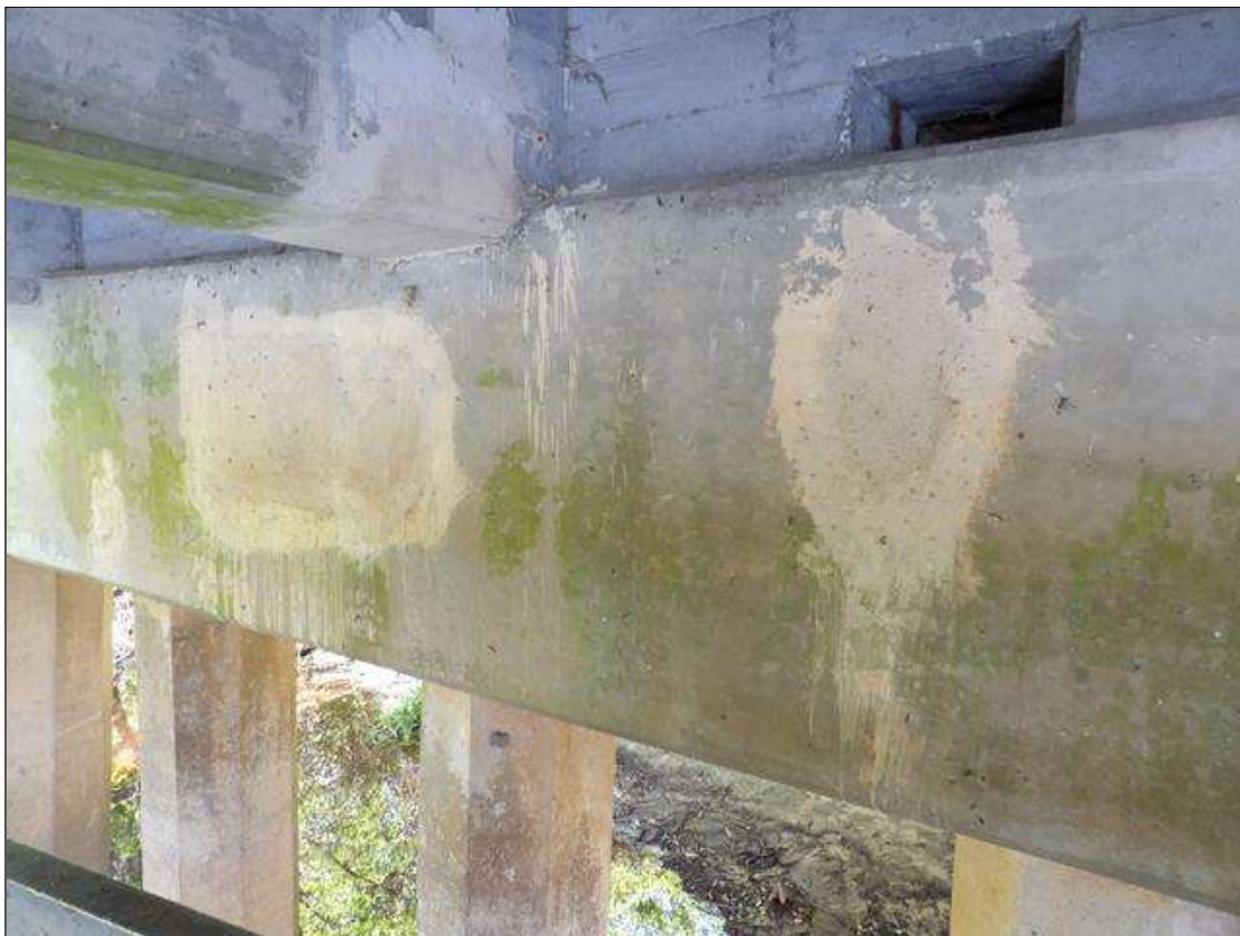
Bent 5 Cap 1: (3) UP TO 3' LONG X 2' HIGH SOUND PATCHES IN WEST FACE AT VARIOUS LOCATIONS
