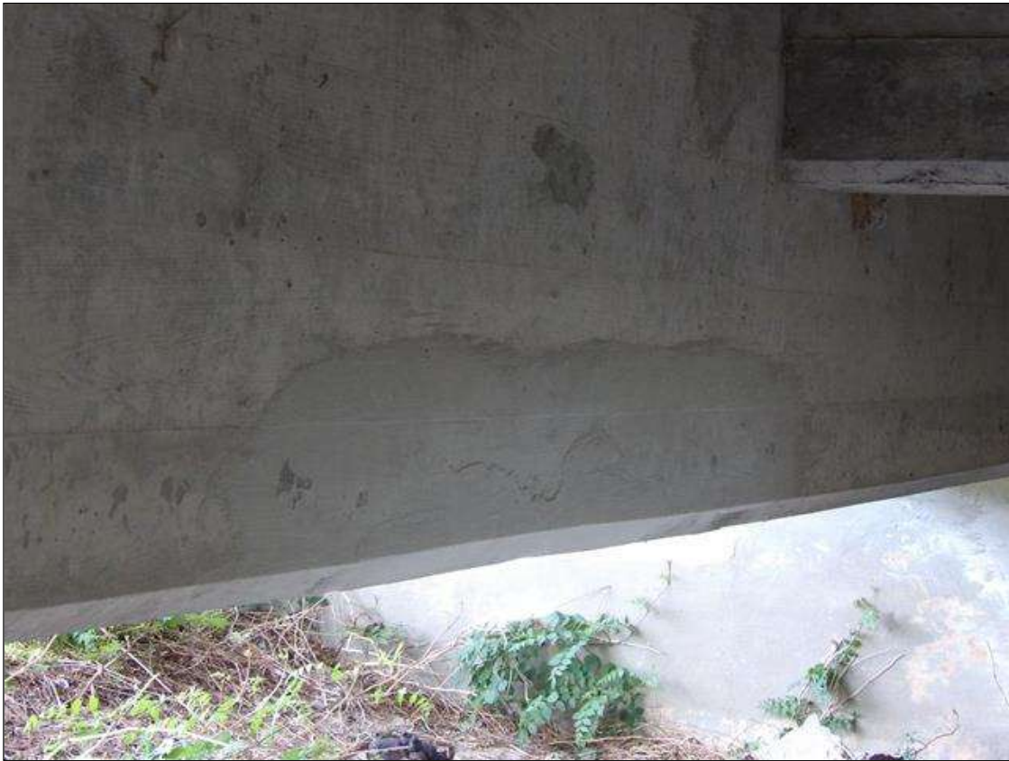
Span 1 Beam 5: 4.5' X 16" AREA PATCH 10' FROM END BENT 1. ON INTERIOR FACE OF WEB EXTENDING ON FULL WIDTH OF BOTTOM FLANGE AND EXTENDING 3" ON EXTERIOR FACE WITH 6" DIAMETER AREA OF DELAMINATION WITH HAIRLINE MAP CRACKING THROUGHOUT PATCH
