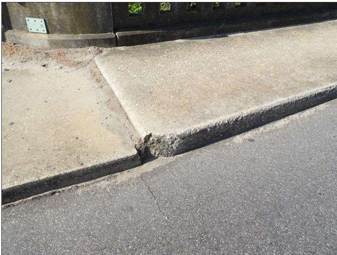
RIGHT SIDEWALK EAST END CORNER SPALL 9" X 7" X UP TO 3" DEEP
