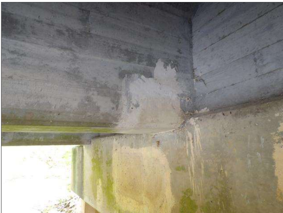
Span 5 Beam 2: 10" LONG X FULL WIDTH SOUND PATCH ON BOTTOM FLANGE AT BENT 5
