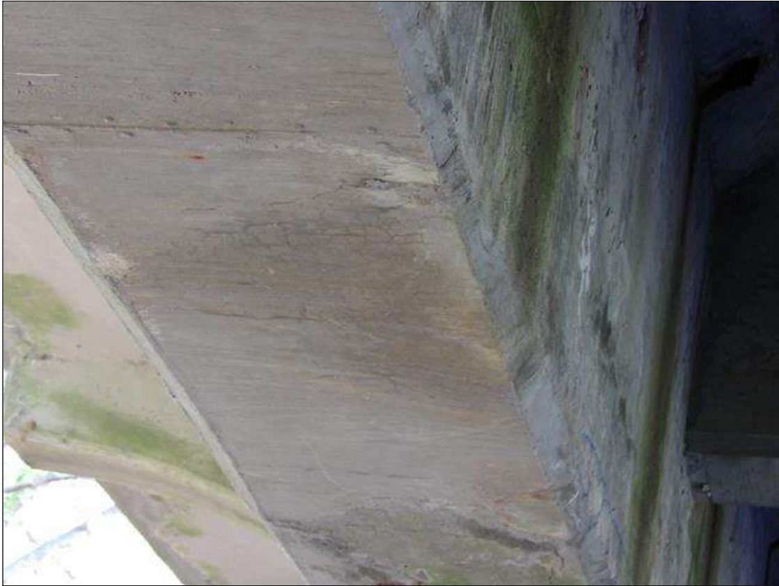
Span 2 Beam 1: SOUND PATCHED AREAS ON THE BOTTOM OF THE BEAM INTERMITTENT THROUGHOUT SPAN EXTENDING 16" FROM BOTTOM OF BEAM ON INTERIOR AND EXTERIOR FACES
