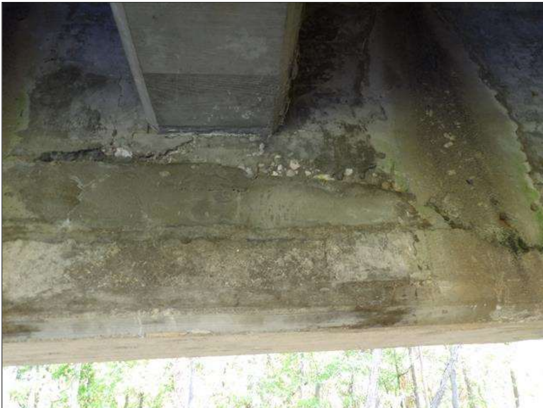
Span 2 Beam 1: PATCHED AREAS ON BOTH FACES THROUGHOUT THE LENGTH OF THE BEAM ARE BEGINNING TO FAIL AND SHOW DELAMINATION
