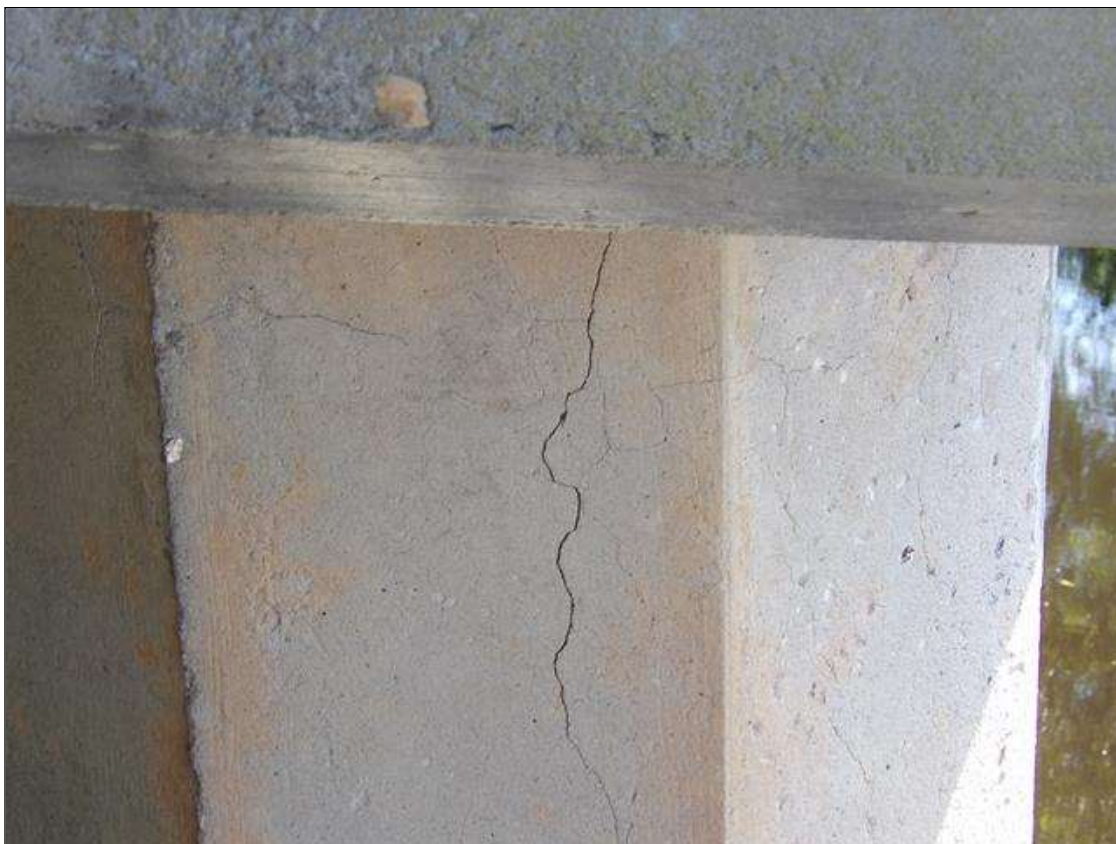
Bent 4 Pile 8: 1' LONG X 1/16" WIDE VERTICAL CRACK IN WEST FACE OF PILE AT CAP
