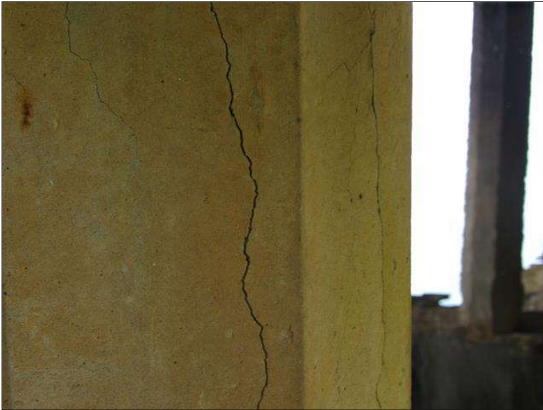
Bent 4 Pile 4: (2) UP TO 2' LONG X 1/16" WIDE VERTICAL CRACKS IN NORTH AND NORTHEAST FACE OF PILE AT TOP
