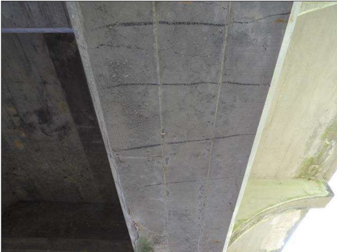
Span 6 Beam 1: 18' LONG X FULL WIDTH AREA OF DELAMINATION IN BOTTOM FLANGE EXTENDING UP TO 1' ON BOTH FACES OF WEB STARTING 10' FROM END BENT 2
