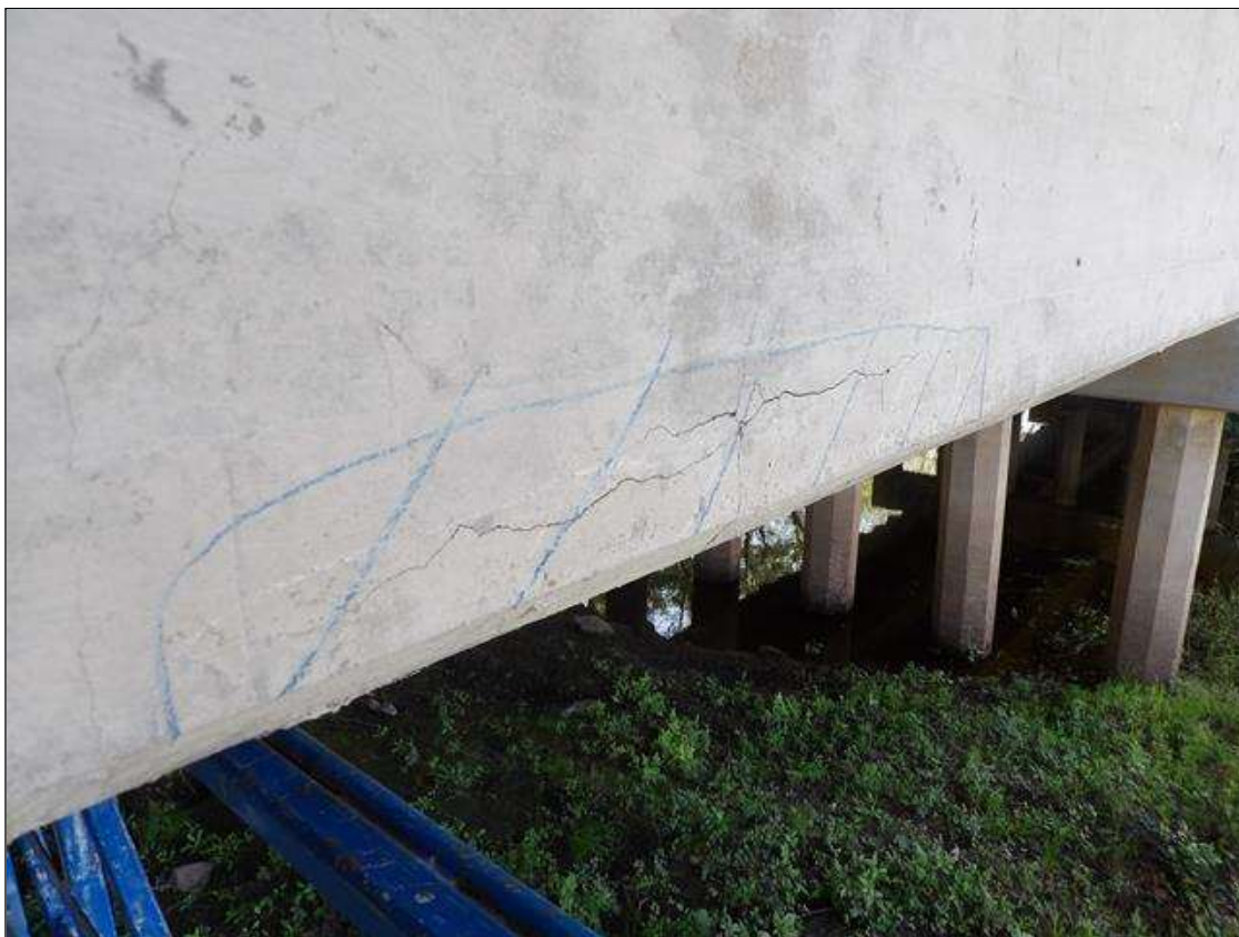
Span 1 Beam 5: 21' FROM END BENT 1, RIGHT SIDE 20" LONG X 3" DELAMINATION
