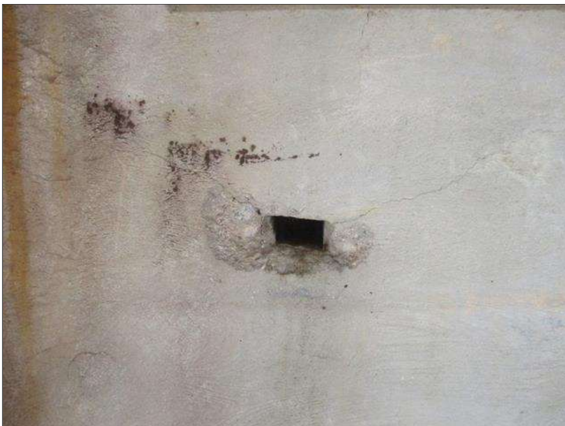
Bent 4 Cap 1: 6" X 4" X 1" DEEP SPALL ON SOUTH FACE UNDER BAY 4
