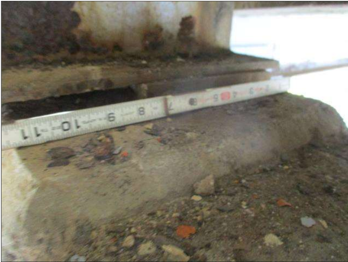
Span 3 Beam 2: [PROMPT ACTION REQUEST] APPROXIMATELY 8" OUT FROM THE BEAM END AT BENT 4, LOWER FLANGE, CORROSION WITH APPROXIMATELY 1/8" SECTION LOSS [AVERAGE 1/4" REMAINS] FOR APPROXIMATELY 4" LONG
