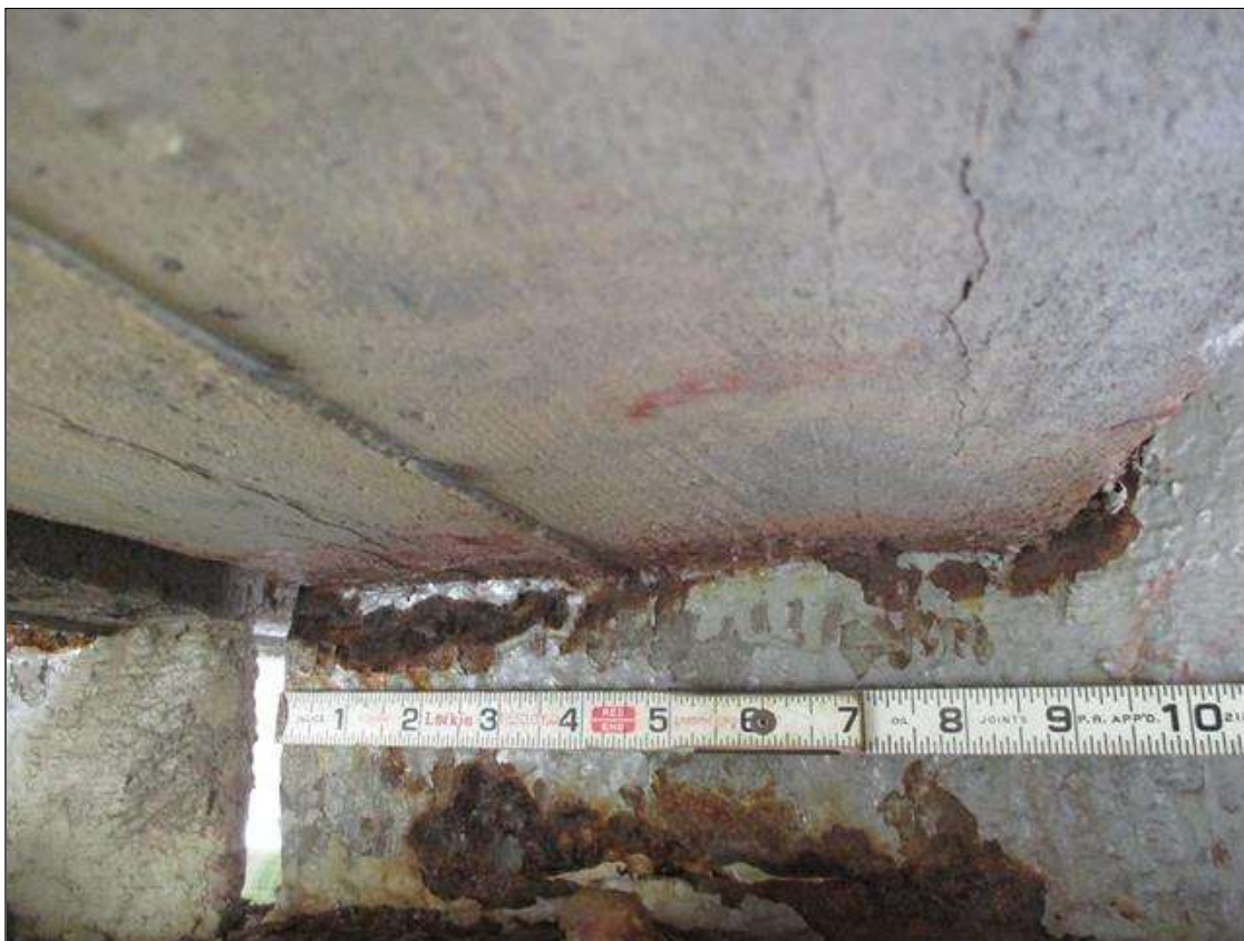
Span 1 Beam 5: [PROMPT ACTION REQUEST] BEAM END AT BENT 2, THERE IS AN APPROXIMATELY 1" WIDE BAND OF CORROSION THAT WRAPS THE REINFORCED CONCRETE DIAPHRAGM, APPROXIMATELY 3/16" SECTION LOSS [AVERAGE 1/8" REMAINS] FOR APPROXIMATELY 3" LONG.
