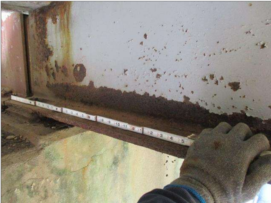
Span 6 Beam 2: [PROMPT ACTION REQUEST] BEAM END AT BENT 5, IN THE LOWER 3" OF THE WEB, CORROSION WITH APPROXIMATELY 1/8" SECTION LOSS [AVERAGE 5/16" REMAINS] FOR 30" LONG.
