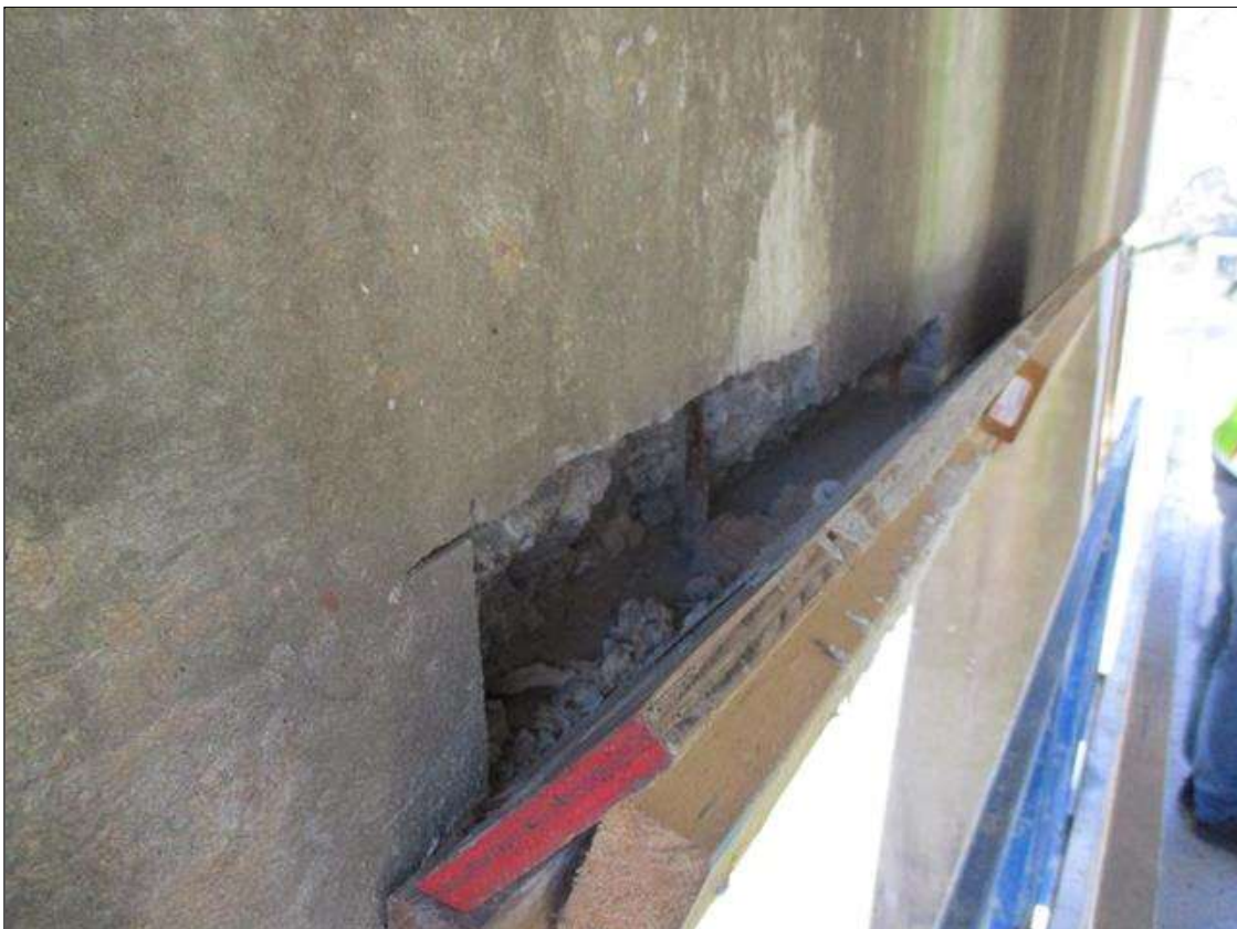
Bent 5 Cap 1: 2.67' X 9" X 5 1/2" DEEP SPALL WITH EXPOSED REBAR ON SOUTH FACE
