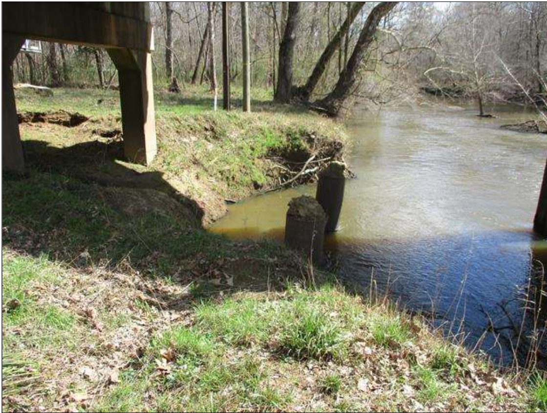
THE SOUTH AND NORTH BANKS HAVE EROSION WITH SLOUGHING [SOUTH APPROXIMATELY 100' LONG X UP TO 10' WIDE X UP TO 10' DEEP, AND NORTH APPROXIMATELY 50' LONG X UP TO 40' WIDE X UP TO 10' DEEP]
