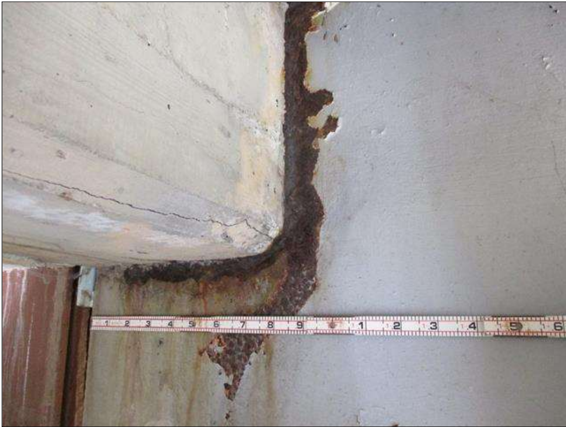
Span 6 Beam 3: [PROMPT ACTION REQUEST] BEAM END AT BENT 5, THERE IS AN APPROXIMATELY 1" WIDE BAND OF CORROSION THAT WRAPS THE REINFORCED CONCRETE DIAPHRAGM, APPROXIMATELY 1/4" SECTION LOSS [AVERAGE 3/16" REMAINS] FOR APPROXIMATELY 10" LONG.
