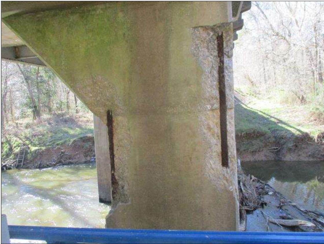
Bent 6 Pile 1: [PROMPT ACTION REQUEST] 2 - UP TO 3' X 10" X 2" DEEP SPALL WITH EXPOSED REBAR ON NORTH FACE [NO MEASURABLE SECTION LOSS]
