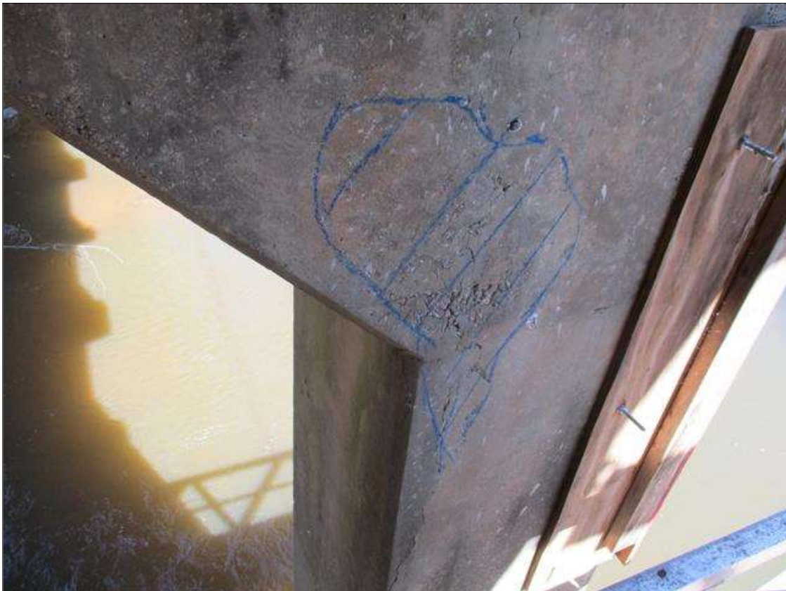
Bent 5 Pile 2: AT THE HAUNCH, APPROXIMATELY 3 SQUARE FEET MAP CRACKING TO 1/16" WIDE AND VERTICAL CRACKING TO 1/8" WIDE WITH ASSOCIATED DELAMINATION
