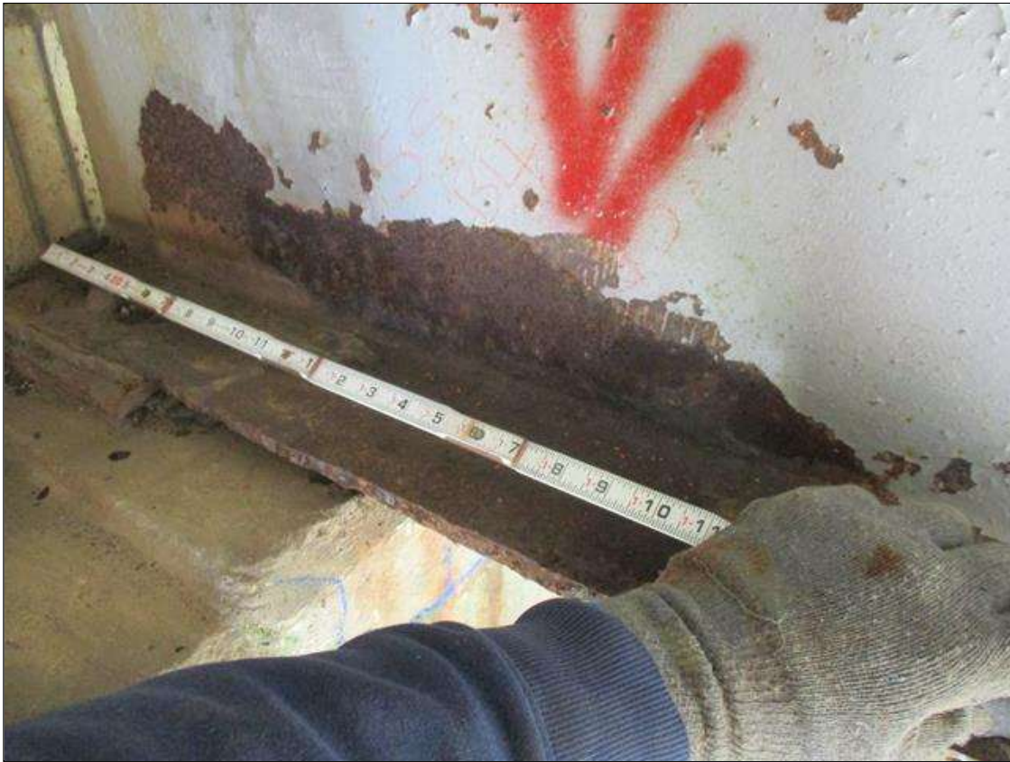
Span 5 Beam 3: [PROMPT ACTION REQUEST] 8" OUT FROM THE BEAM END AT BENT 4, IN THE LOWER 2" OF THE WEB, CORROSION WITH APPROXIMATELY 3/16" SECTION LOSS [AVERAGE 1/4" REMAINS] FOR 12" LONG.
