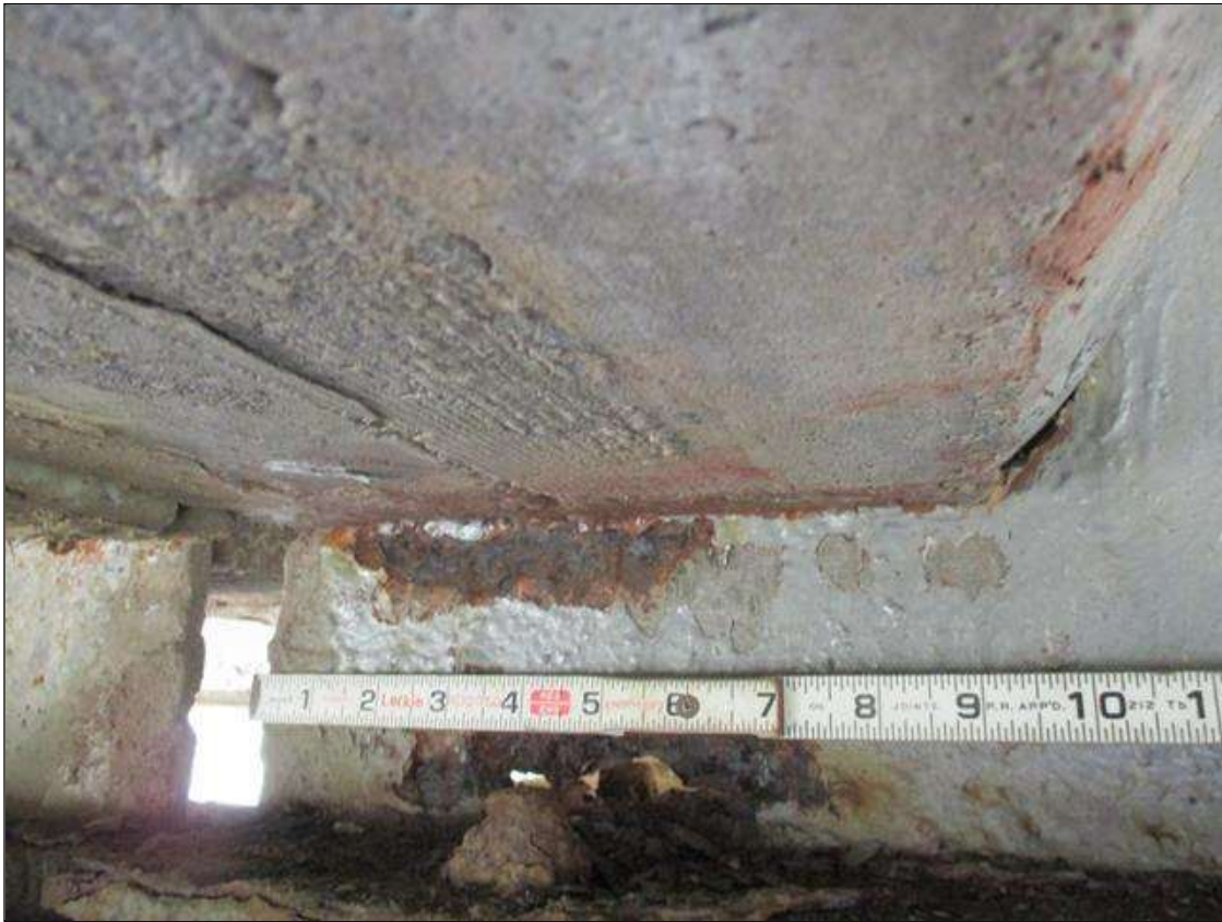
Span 1 Beam 3: [PROMPT ACTION REQUEST] BEAM END AT BENT 2, THERE IS AN APPROXIMATELY 1" WIDE BAND OF CORROSION THAT WRAPS THE REINFORCED CONCRETE DIAPHRAGM, APPROXIMATELY 3/16" SECTION LOSS [AVERAGE 1/8" REMAINS] FOR APPROXIMATELY 5" LONG.
