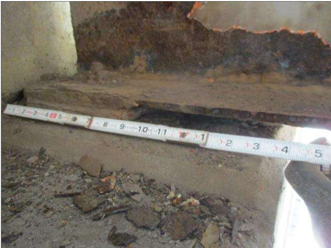
Span 8 Beam 3: [PROMPT ACTION REQUEST] BEAM END AT BENT 8, LOWER FLANGE, CORROSION WITH APPROXIMATELY 5/16" SECTION LOSS [AVERAGE 5/16" REMAINS] FOR APPROXIMATELY 1.5' LONG.
