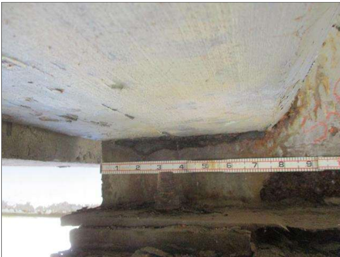
Span 3 Beam 3: [PROMPT ACTION REQUEST] APPROXIMATELY 1" OUT FROM THE BEAM END AT BENT 4, THERE IS AN APPROXIMATELY 1" WIDE BAND OF CORROSION THAT WRAPS THE REINFORCED CONCRETE DIAPHRAGM, APPROXIMATELY 3/16" SECTION LOSS [AVERAGE 1/8" REMAINS] FOR APPROXIMATELY 9" LONG.
