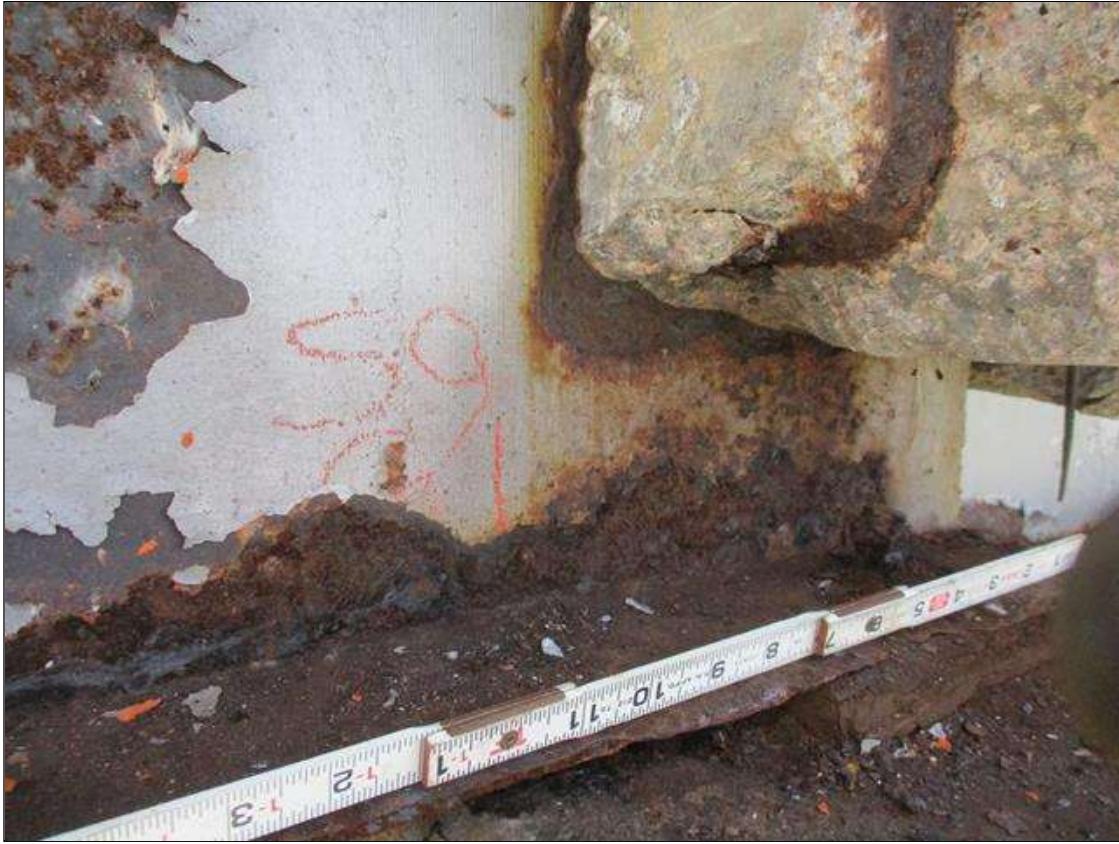
Span 9 Beam 1: [PROMPT ACTION REQUEST] BEAM END AT BENT 8, WEB, LOWER 2", CORROSION WITH APPROXIMATELY 1/8" SECTION LOSS [AVERAGE 1/4" REMAINS] FOR 12" LONG
