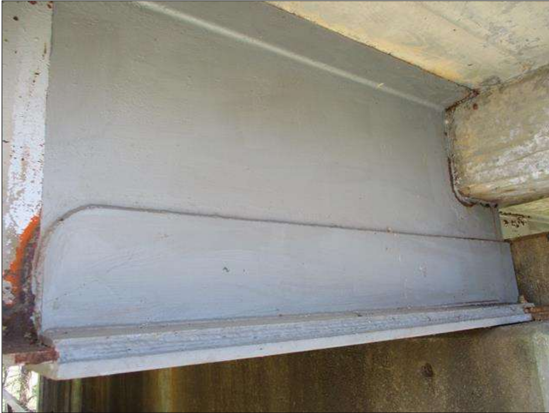
Span 5 Beam 1: [NEW REPAIR] BEAM END AT BENT 4, PLATES HAVE BEEN WELDED TO BOTH SIDES OF THE WEB [4.67' LONG X 6" HIGH] AND ON THE UPPER AND LOWER SIDES OF THE LOWER FLANGE [4.67' LONG X 1' WIDE] IN THE AREAS OF PAST SECTION LOSS.
