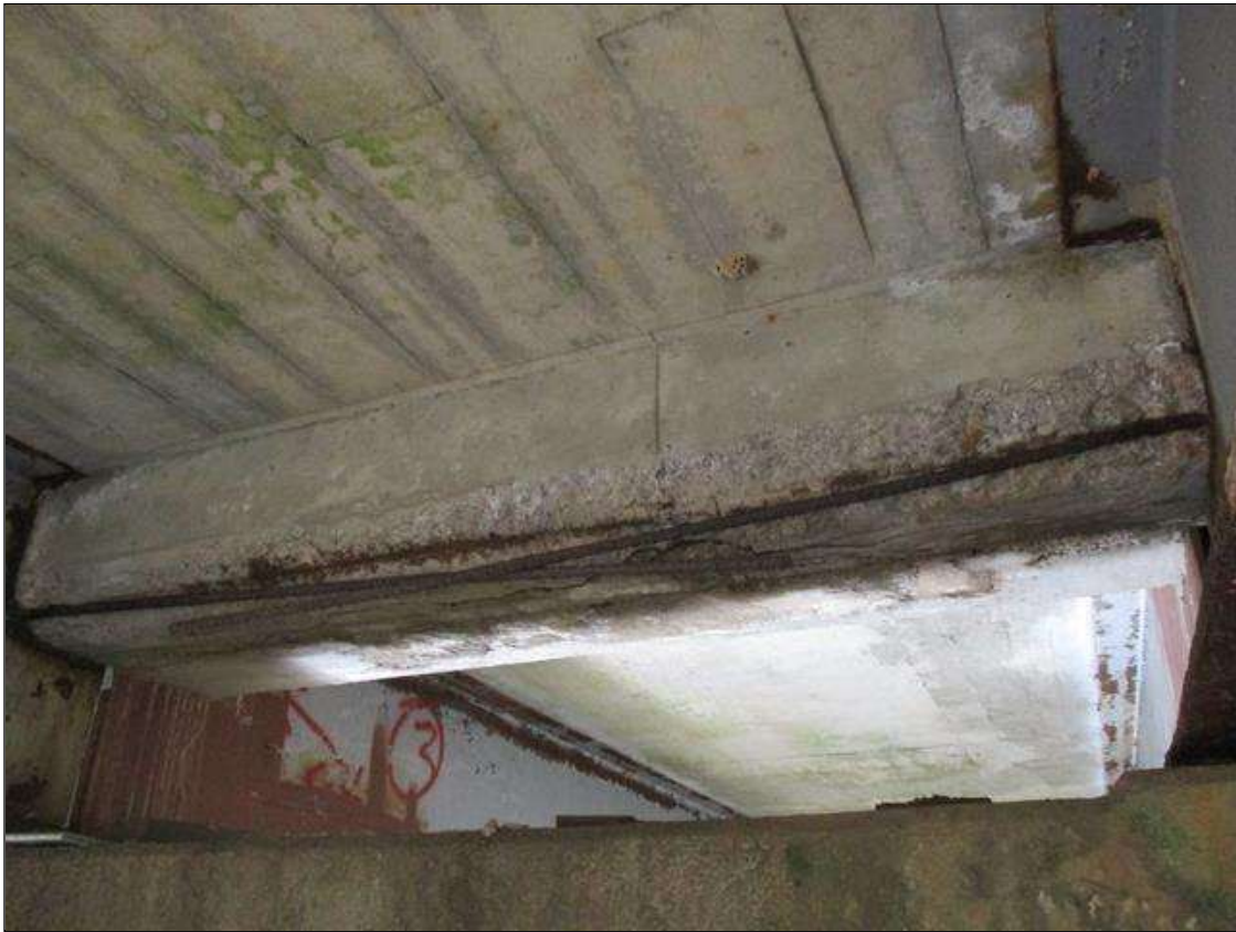
Span 6 Beam 2: [PROMPT ACTION REQUEST] BAY 2 AT BENT 5, REINFORCED CONCRETE DIAPHRAGM, SPALLING WITH EXPOSED REBAR [APPROXIMATELY 6' LONG X 12" WIDE X UP TO 2" DEEP] WITH DELAMINATED REBAR, WHICH HAS SURFACE CORROSION AND PITTING UP TO 1/8" DEEP
