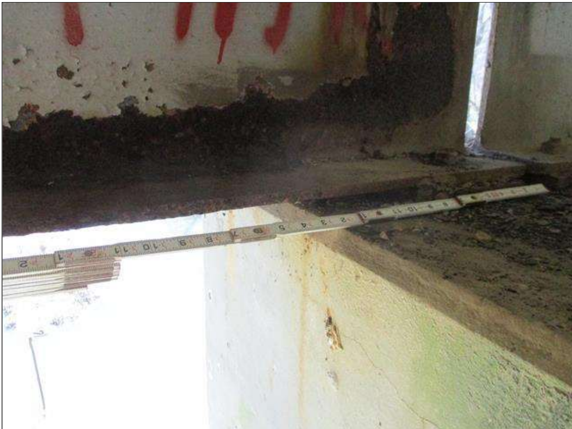
Span 7 Beam 4: [PROMPT ACTION REQUEST] BEAM END AT BENT 6, LOWER FLANGE, CORROSION WITH APPROXIMATELY 3/16" SECTION LOSS [AVERAGE 7/16" REMAINS] FOR APPROXIMATELY 12" LONG
