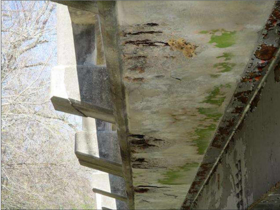
REINFORCED CONCRETE DECK OVERHANGS: VIEW OF TYPICAL SCATTERED SPALLING WITH EXPOSED REBAR AND DELAMINATION
