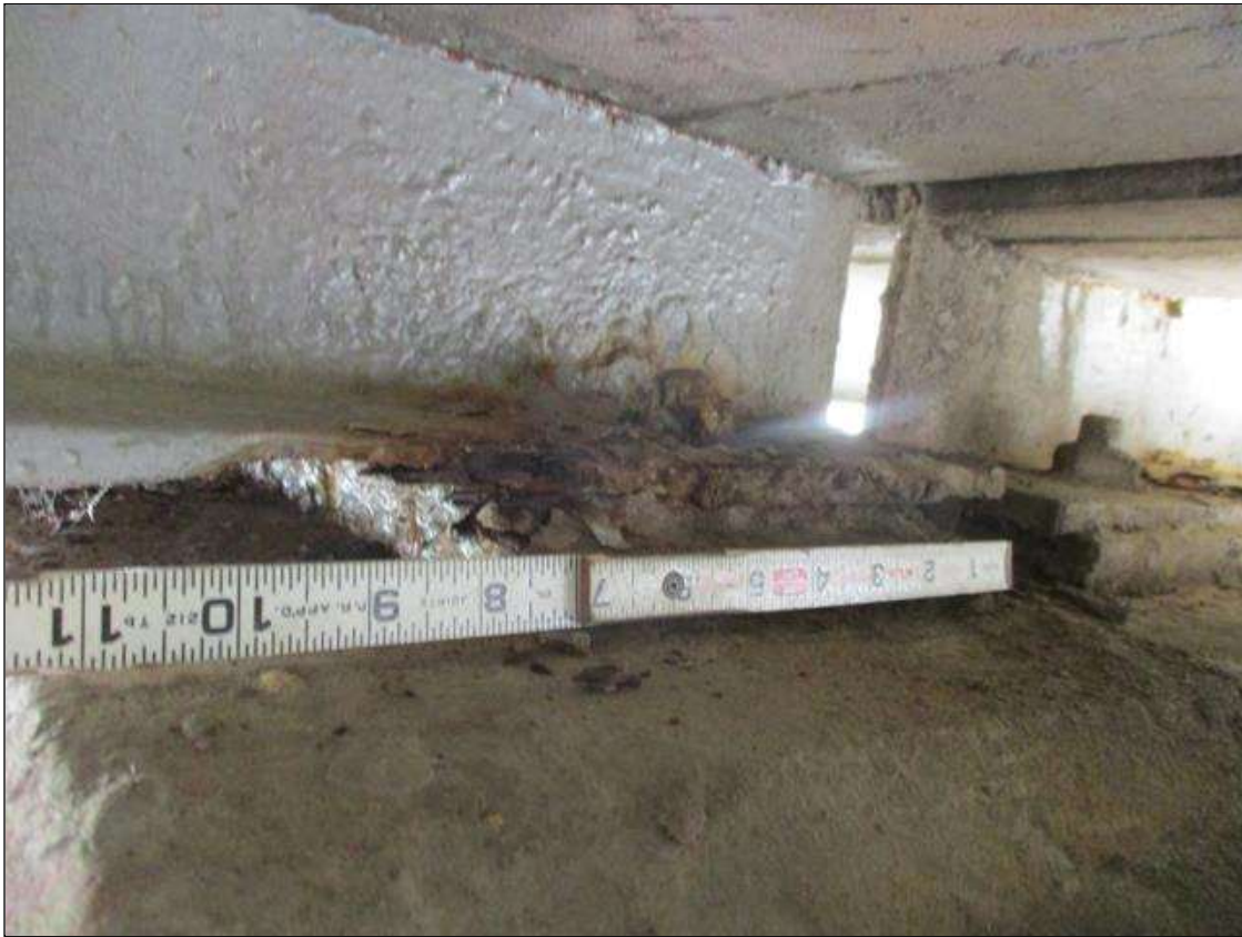
Span 1 Beam 2: [PROMPT ACTION REQUEST] APPROXIMATELY 6" OUT FROM THE BEAM END AT BENT 2, LOWER FLANGE, CORROSION WITH APPROXIMATELY 3/16" SECTION LOSS [AVERAGE 3/16" REMAINS] FOR APPROXIMATELY 3" LONG
