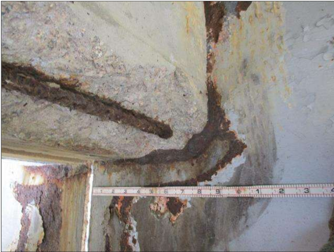
Span 7 Beam 1: [PROMPT ACTION REQUEST] BEAM END AT BENT 6, THERE IS AN APPROXIMATELY 1" WIDE BAND OF CORROSION THAT WRAPS THE REINFORCED CONCRETE DIAPHRAGM, APPROXIMATELY 3/16" SECTION LOSS [AVERAGE 1/4" REMAINS] FOR APPROXIMATELY 10" LONG.
