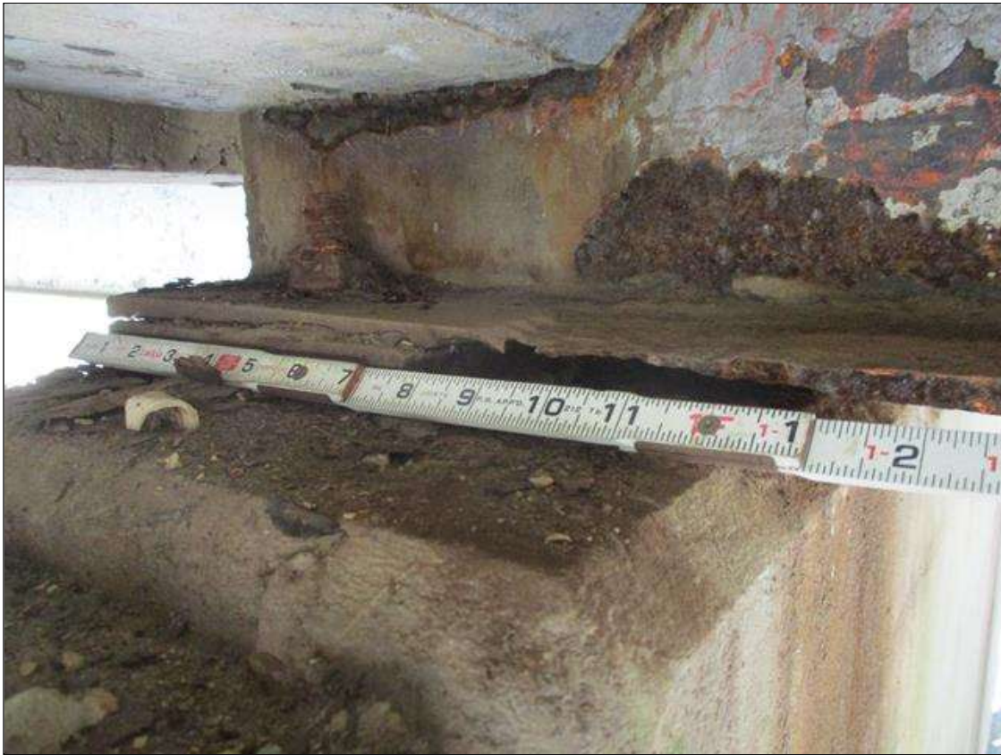
Span 3 Beam 3: [PROMPT ACTION REQUEST] BEAM END AT BENT 4, LOWER FLANGE, CORROSION WITH APPROXIMATELY 1/4" SECTION LOSS [AVERAGE 1/8" REMAINS] FOR APPROXIMATELY 12" LONG
