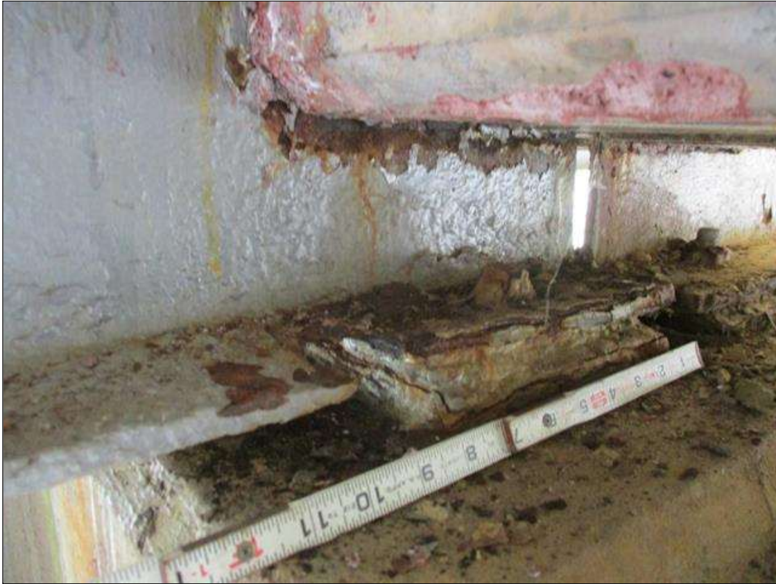
Span 1 Beam 4: [PROMPT ACTION REQUEST] BEAM END AT BENT 2, LOWER LEFT FLANGE, CORROSION WITH APPROXIMATELY 1/4" SECTION LOSS [AVERAGE 1/8" REMAINS] FOR APPROXIMATELY 11" LONG, AND LOWER RIGHT FLANGE, CORROSION WITH 100% SECTION LOSS FOR APPROXIMATELY 11" LONG
