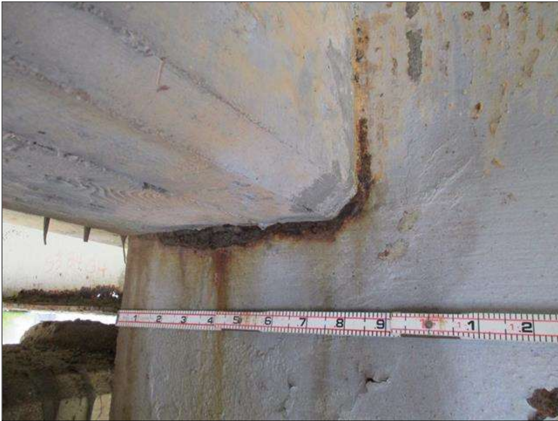
Span 5 Beam 2: [PROMPT ACTION REQUEST] BEAM END AT BENT 4, THERE IS AN APPROXIMATELY 1" WIDE BAND OF CORROSION THAT WRAPS THE REINFORCED CONCRETE DIAPHRAGM, APPROXIMATELY 1/8" SECTION LOSS [AVERAGE 5/16" REMAINS] FOR APPROXIMATELY 10" LONG.
