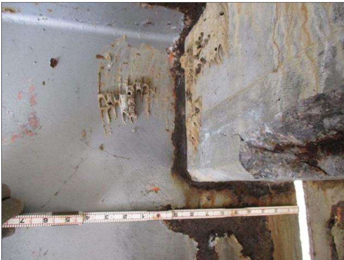
Span 5 Beam 1: [PROMPT ACTION REQUEST] BEAM END AT BENT 5, THERE IS AN APPROXIMATELY 1" WIDE BAND OF CORROSION THAT WRAPS THE REINFORCED CONCRETE DIAPHRAGM, APPROXIMATELY 1/4" SECTION LOSS [AVERAGE 3/16" REMAINS] FOR APPROXIMATELY 10" LONG.
