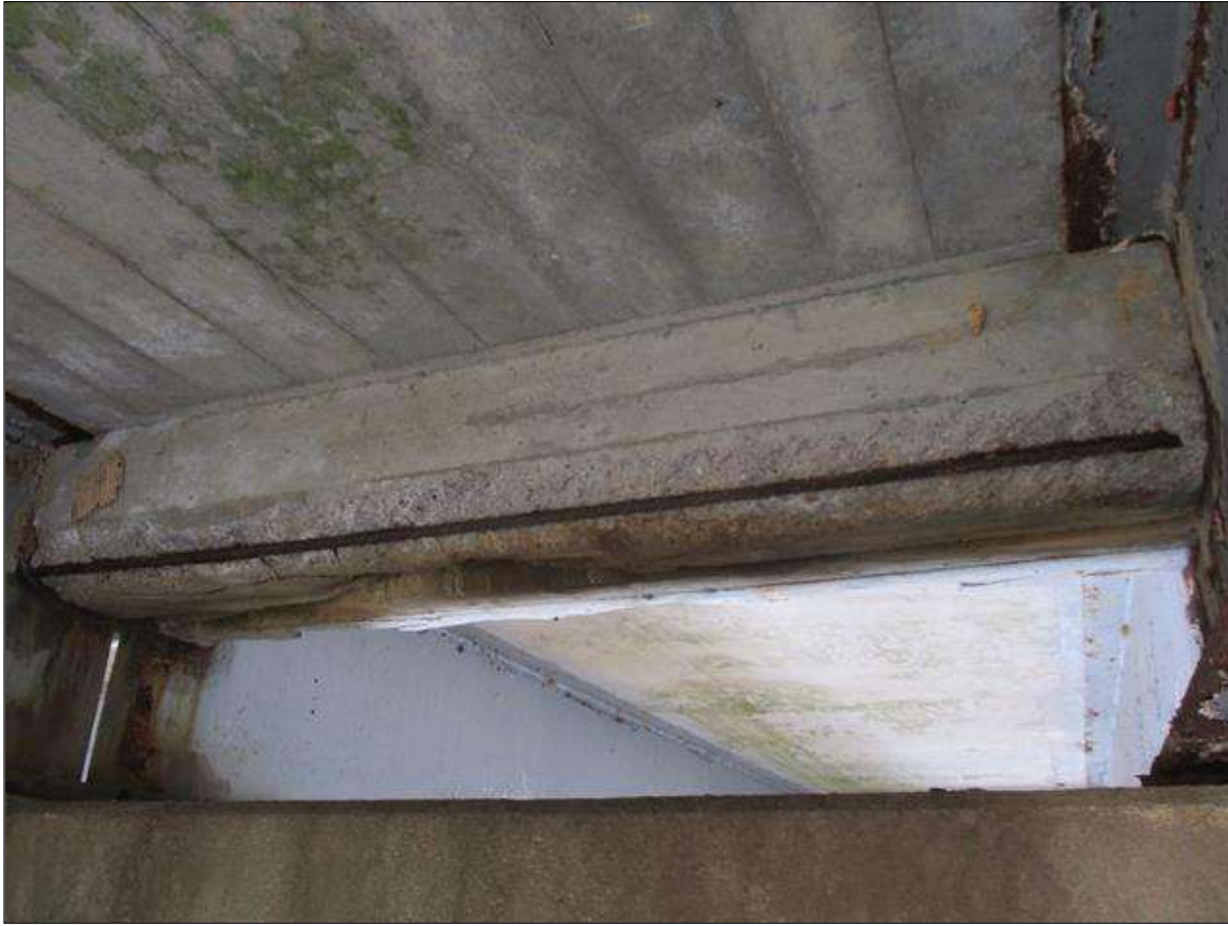
Span 7 Beam 1: [PROMPT ACTION REQUEST] BAY 1 AT BENT 6, REINFORCED CONCRETE DIAPHRAGM, SPALLING WITH EXPOSED REBAR [APPROXIMATELY 6' LONG X 12" WIDE X UP TO 2" DEEP] WITH DELAMINATED REBAR, WHICH HAS SURFACE CORROSION AND PITTING UP TO 1/8" DEEP
