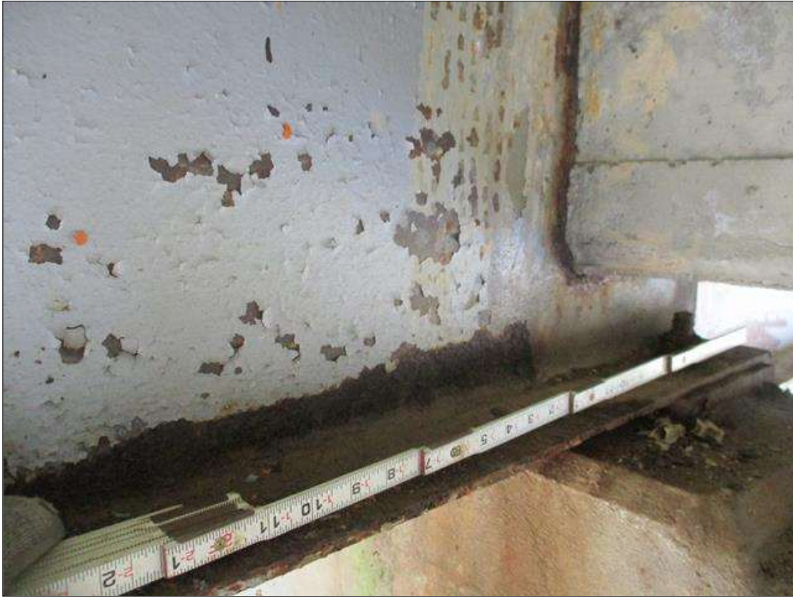
Span 3 Beam 3: [PROMPT ACTION REQUEST] APPROXIMATELY 10" OUT FROM THE BEAM END AT BENT 4, IN THE LOWER 2" OF THE WEB, CORROSION WITH APPROXIMATELY 1/8" SECTION LOSS [AVERAGE 3/16" REMAINS] FOR APPROXIMATELY 12" LONG.
