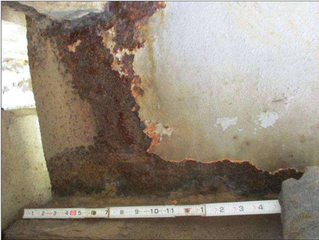
Span 8 Beam 3: [PROMPT ACTION REQUEST] BEAM END AT BENT 8, WEB, FULL HEIGHT, CORROSION WITH APPROXIMATELY 3/16" SECTION LOSS [AVERAGE 1/4" REMAINS] FOR 10" LONG
