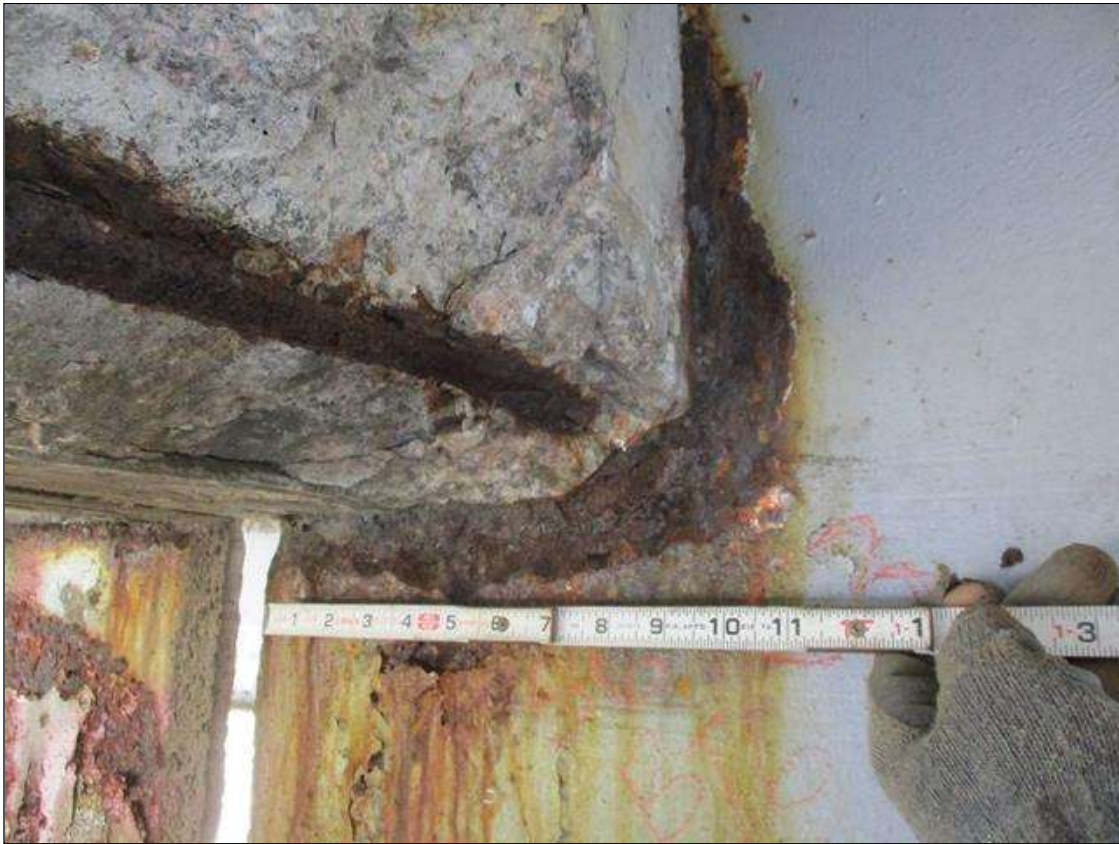
Span 5 Beam 3: [PROMPT ACTION REQUEST] BEAM END AT BENT 5, THERE IS AN APPROXIMATELY 2" WIDE BAND OF CORROSION THAT WRAPS THE REINFORCED CONCRETE DIAPHRAGM, APPROXIMATELY 5/16" SECTION LOSS [AVERAGE 1/8" REMAINS] FOR APPROXIMATELY 10" LONG.
