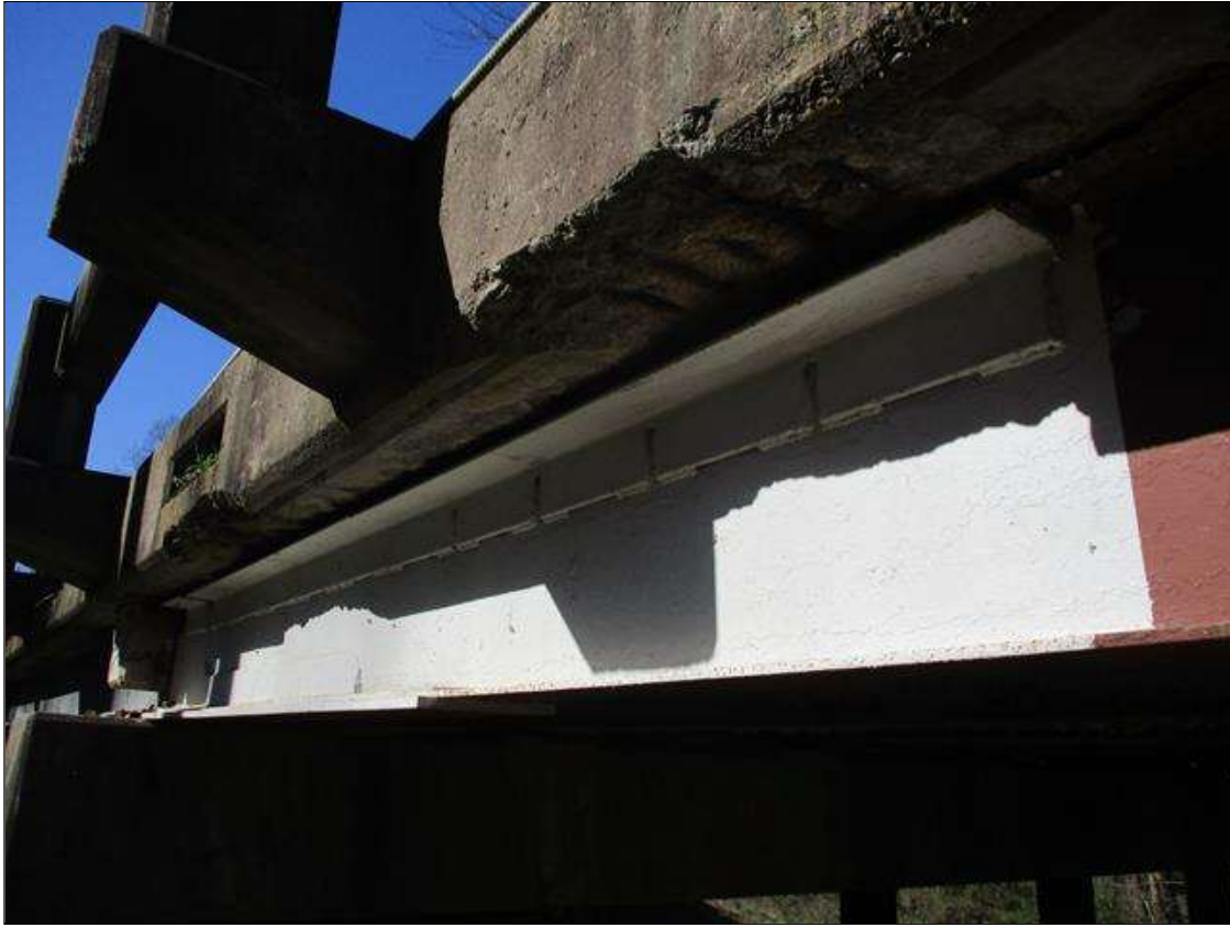
Span 3 Beam 6: [NEW REPAIR] BEAM END AT BENT 2, PLATES HAVE BEEN WELDED TO BOTH SIDES OF THE LOWER WEB [APPROXIMATELY 84" LONG X UP TO 14" HIGH X 3/8" THICK]; AND THE LOWER FLANGE [APPROXIMATELY 91" LONG X 10" WIDE X 3/4" THICK]; AND THE UPPER RIGHT FLANGE [APPROXIMATELY 134" LONG X 4" WIDE]
