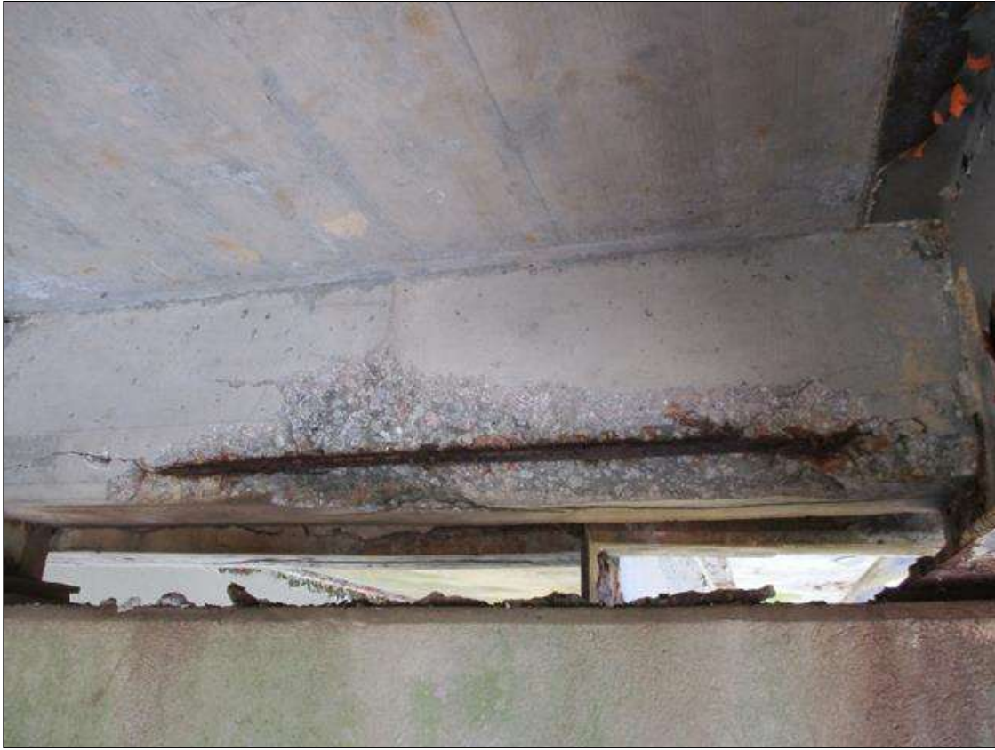
Span 9 Beam 3: [PROMPT ACTION REQUEST] BAY 2 AT BENT 8, REINFORCED CONCRETE DIAPHRAGM, SPALLING WITH EXPOSED REBAR [APPROXIMATELY 4' LONG X 10" WIDE X UP TO 3" DEEP]. THE REBAR IS DELAMINATED FROM THE CONCRETE AND HAS SURFACE CORROSION AND PITTING UP TO 1/16" DEEP.
