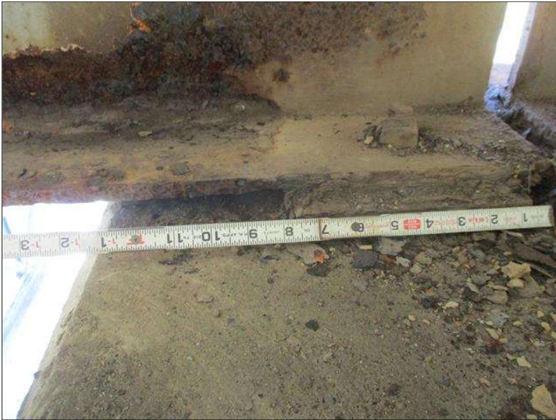
Span 5 Beam 1: [PROMPT ACTION REQUEST] BEAM END AT BENT 5, LOWER FLANGE, CORROSION WITH APPROXIMATELY 3/16" SECTION LOSS [AVERAGE 7/16" REMAINS] FOR APPROXIMATELY 10" LONG
