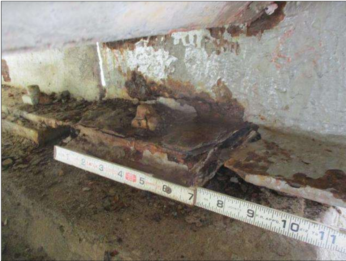
Span 1 Beam 5: [PROMPT ACTION REQUEST] BEAM END AT BENT 2, LOWER FLANGE, CORROSION WITH 100% SECTION LOSS FOR APPROXIMATELY 8" LONG
