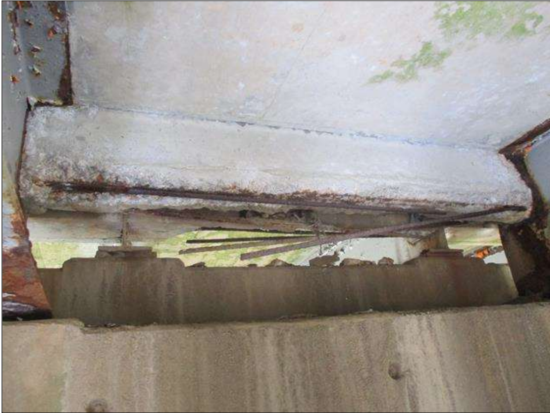
Span 8 Beam 2: [PROMPT ACTION REQUEST] BAY 2 AT BENT 8, REINFORCED CONCRETE DIAPHRAGM, SPALLING WITH EXPOSED REBAR [APPROXIMATELY 6' LONG X 1' WIDE X UP TO 4" DEEP]. THE REBAR IS DELAMINATED FROM THE CONCRETE AND HAS SURFACE CORROSION AND PITTING UP TO 1/16" DEEP.
