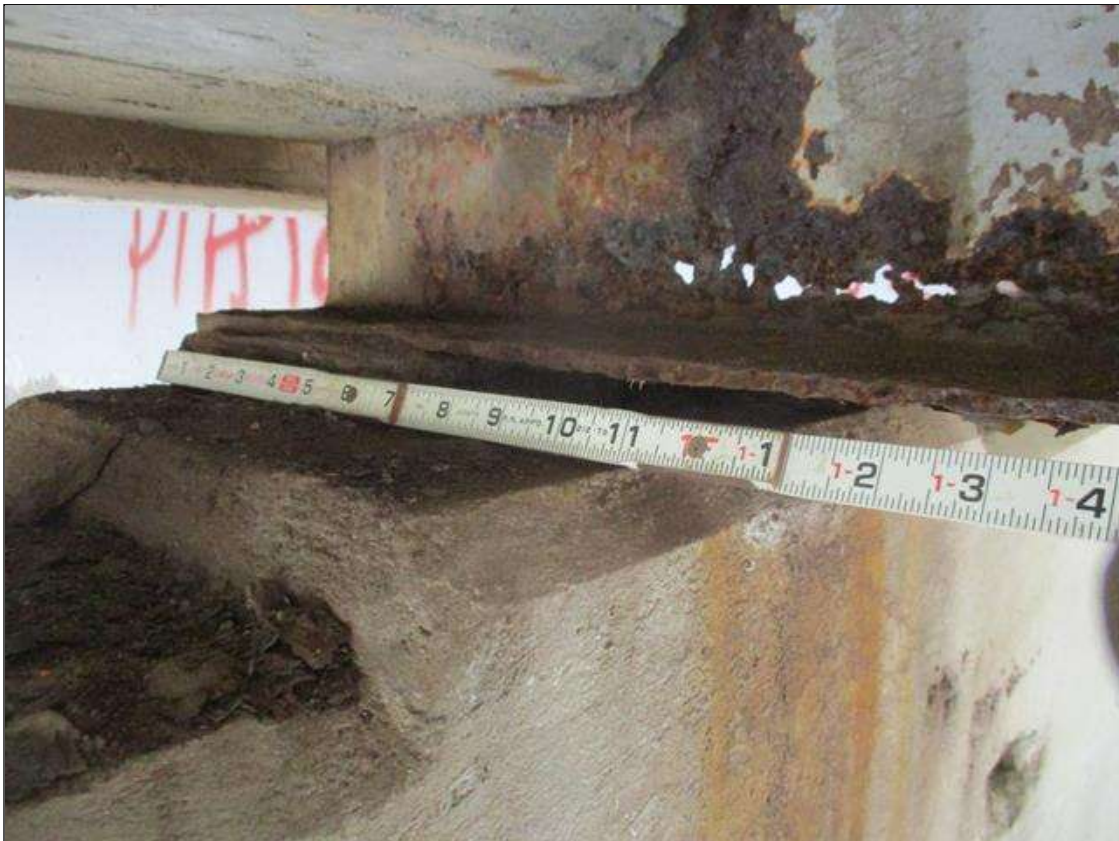
Span 3 Beam 4: [PROMPT ACTION REQUEST] BEAM END AT BENT 4, LOWER FLANGE, CORROSION WITH APPROXIMATELY 3/16" SECTION LOSS [AVERAGE 3/16" REMAINS] FOR APPROXIMATELY 20" LONG
