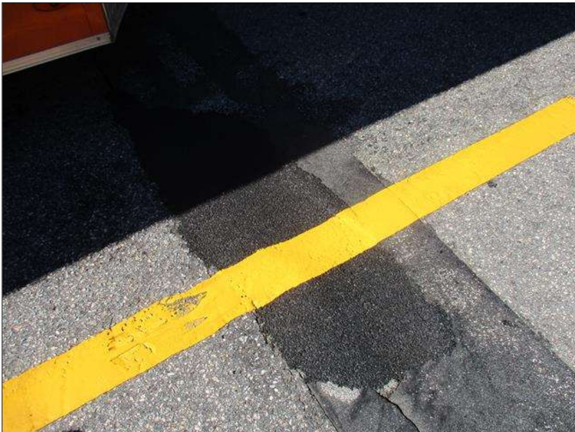
Expansion Joint : SCATTERED 1/2" LONGITUDINAL CRACKING AND APPROXIMATELY 4 SQUARE FEET UNSOUND PATCHING [COLD PATCH]
