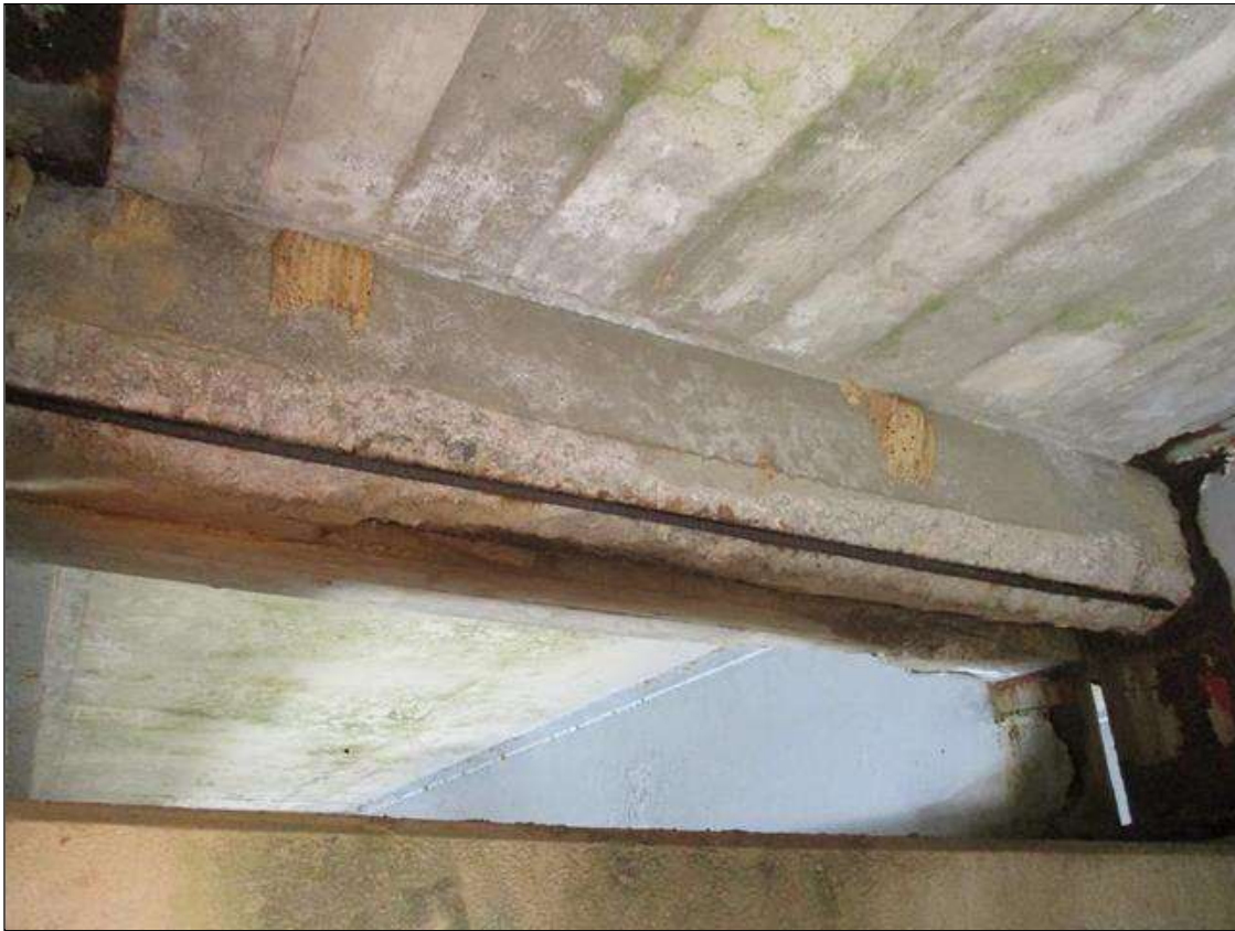
Span 7 Beam 3: [PROMPT ACTION REQUEST] BAY 3 AT BENT 6, REINFORCED CONCRETE DIAPHRAGM, SPALLING WITH EXPOSED REBAR [APPROXIMATELY 6' LONG X 12" WIDE X UP TO 3" DEEP] WITH DELAMINATED REBAR, WHICH HAS SURFACE CORROSION AND PITTING UP TO 1/8" DEEP THROUGHOUT WITH AREAS OF SECTION LOSS UP TO 90%
