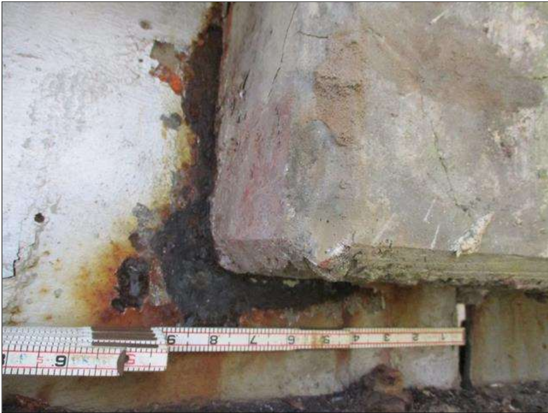
Span 3 Beam 1: [PROMPT ACTION REQUEST] APPROXIMATELY 5" OUT FROM THE BEAM END AT BENT 2, THERE IS AN APPROXIMATELY 1" WIDE BAND OF CORROSION THAT WRAPS THE REINFORCED CONCRETE DIAPHRAGM, 100% SECTION LOSS FOR APPROXIMATELY 5" LONG.
