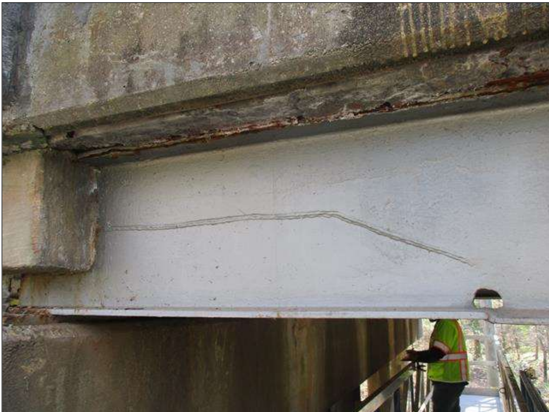
Span 1 Beam 1: [NEW REPAIR] BEAM END AT BENT 2 HAS BEEN SECTIONED, APPROXIMATELY 4' LONG X 7.5" WIDE X UP TO 8" HIGH
