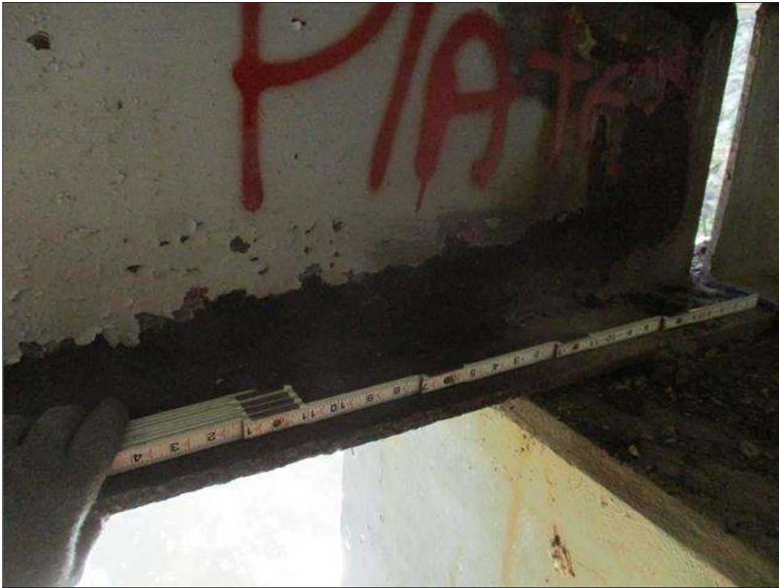
Span 7 Beam 4: [PROMPT ACTION REQUEST] 12" OUT FROM THE BEAM END AT BENT 6, IN THE LOWER 2" OF THE WEB, CORROSION WITH APPROXIMATELY 3/16" SECTION LOSS [AVERAGE 1/4" REMAINS] FOR 18" LONG.
