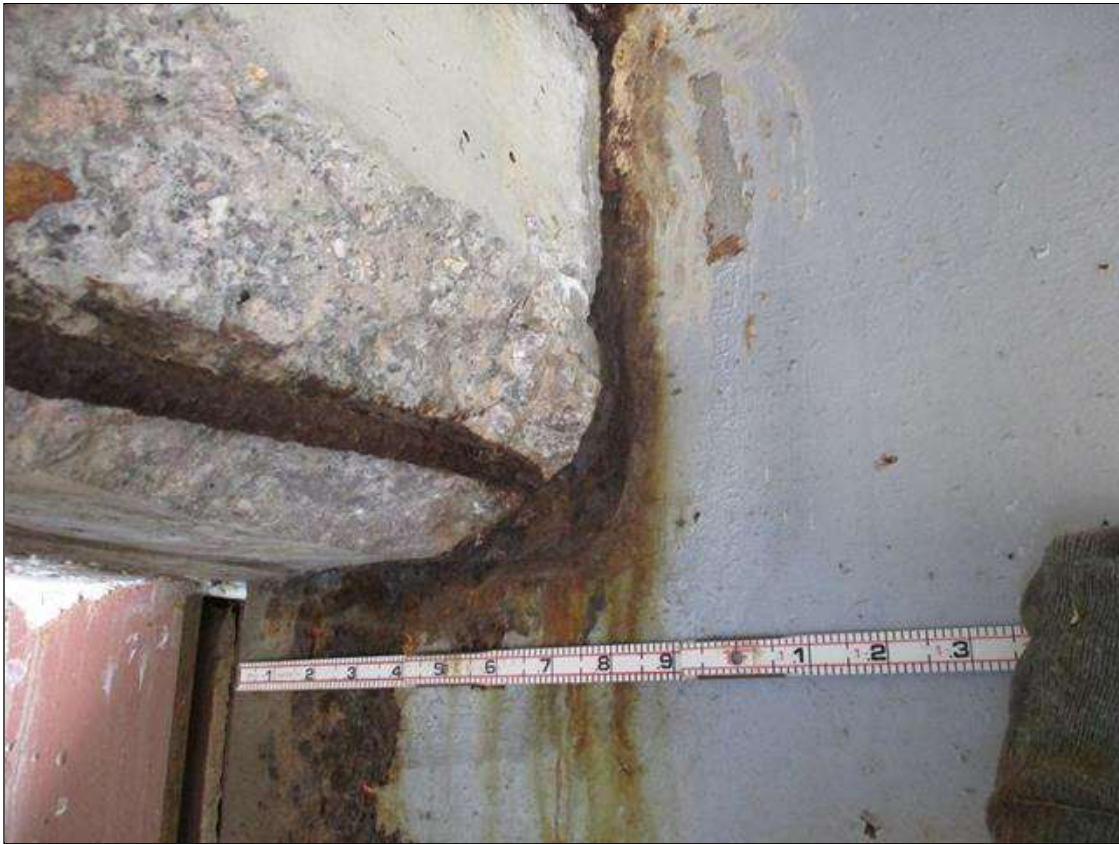
Span 6 Beam 2: [PROMPT ACTION REQUEST] BEAM END AT BENT 5, THERE IS AN APPROXIMATELY 2" WIDE BAND OF CORROSION THAT WRAPS THE REINFORCED CONCRETE DIAPHRAGM, APPROXIMATELY 3/16" SECTION LOSS [AVERAGE 1/4" REMAINS] FOR APPROXIMATELY 10" LONG.
