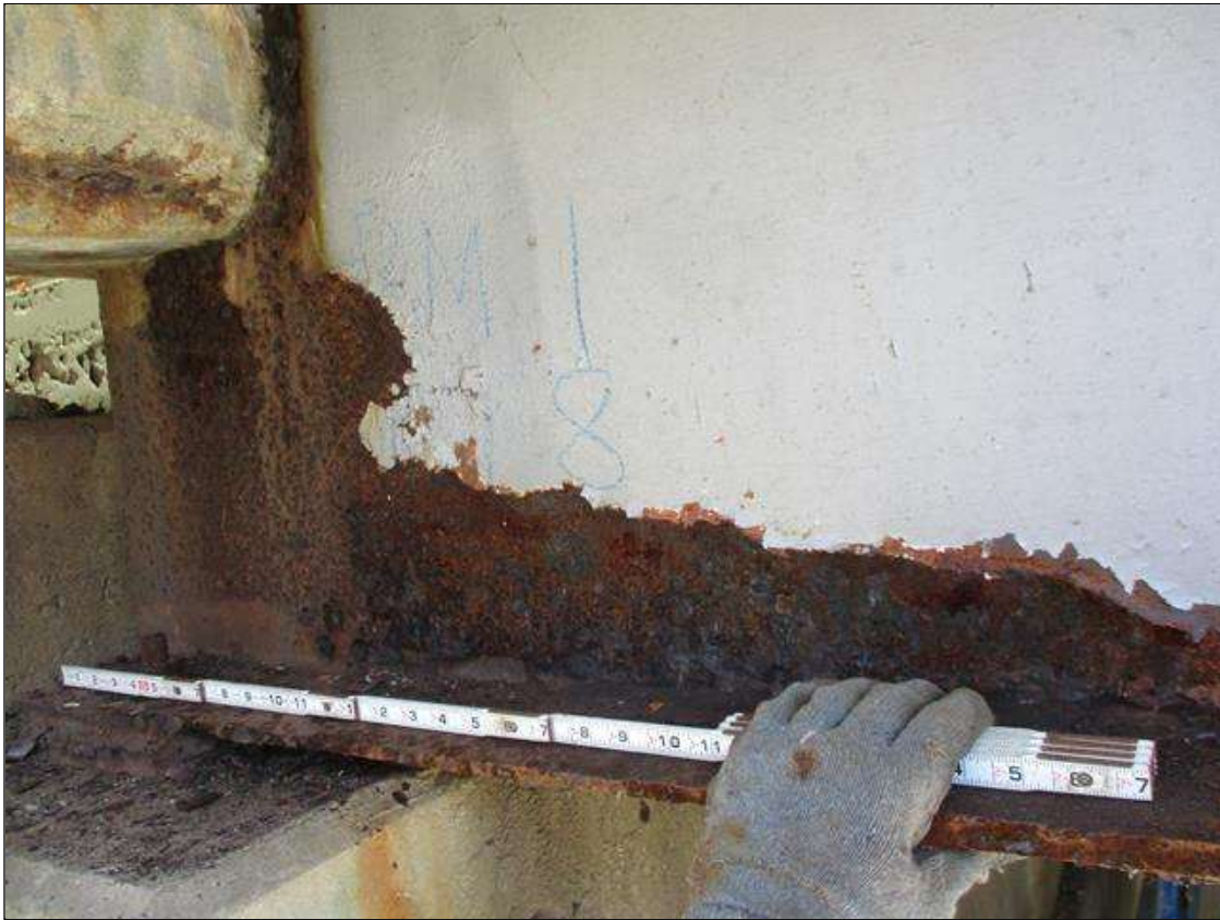
Span 8 Beam 1: [PROMPT ACTION REQUEST] BEAM END AT BENT 8, WEB, FULL HEIGHT, CORROSION WITH APPROXIMATELY 1/8" SECTION LOSS [AVERAGE 5/16" REMAINS] FOR 10" LONG, THEN IN THE LOWER 5" OF THE WEB, CORROSION WITH APPROXIMATELY 1/8" SECTION LOSS [AVERAGE 5/16" REMAINS] FOR 18" LONG.
