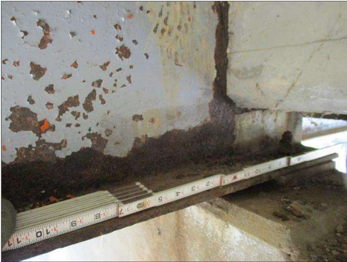
Span 3 Beam 2: [PROMPT ACTION REQUEST] APPROXIMATELY 10" OUT FROM THE BEAM END AT BENT 4, IN THE LOWER 1" OF THE WEB, CORROSION WITH APPROXIMATELY 1/8" SECTION LOSS [AVERAGE 3/16" REMAINS] FOR APPROXIMATELY 15" LONG.
