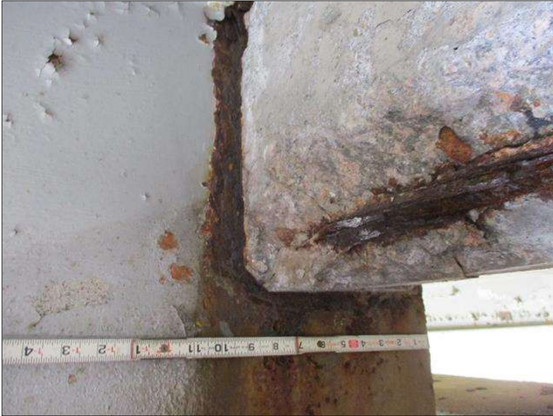
Span 8 Beam 2: [PROMPT ACTION REQUEST] BEAM END AT BENT 8, THERE IS AN APPROXIMATELY 1" WIDE BAND OF CORROSION THAT WRAPS THE REINFORCED CONCRETE DIAPHRAGM, APPROXIMATELY 3/16" SECTION LOSS [AVERAGE 1/4" REMAINS] FOR APPROXIMATELY 10" LONG.
