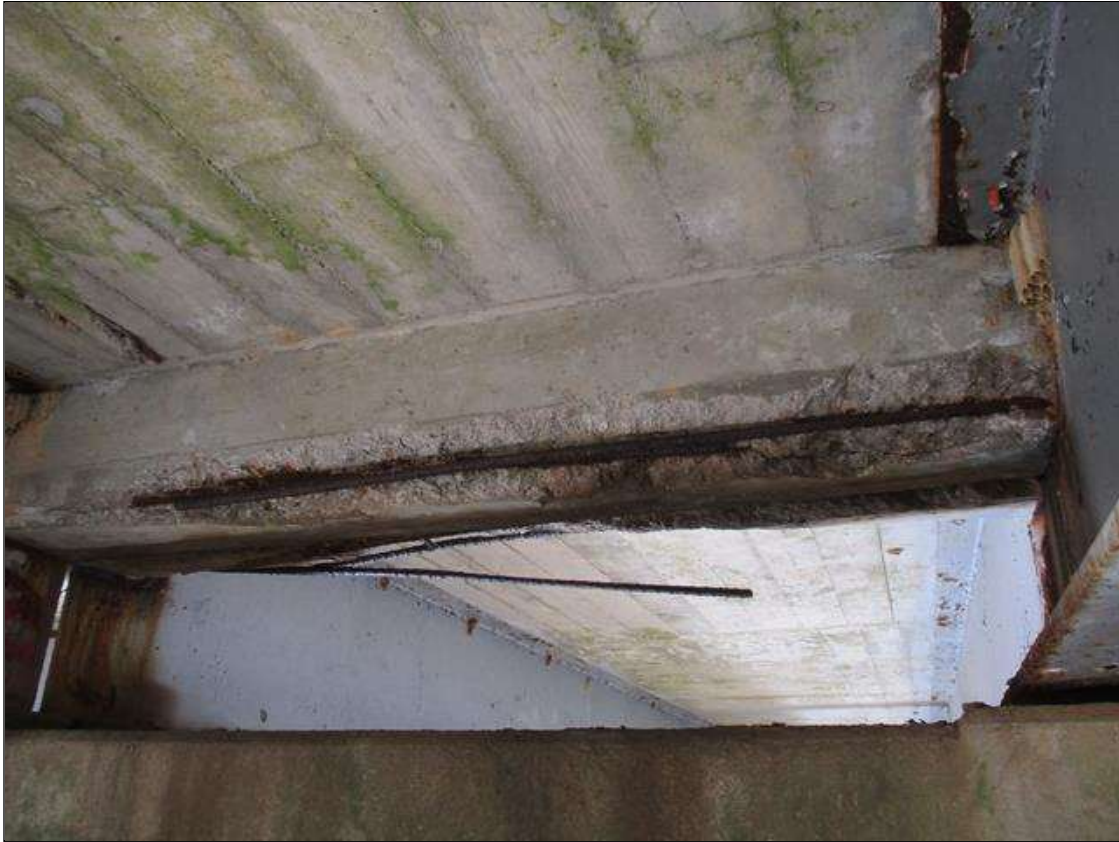
Span 7 Beam 2: [PROMPT ACTION REQUEST] BAY 2 AT BENT 6, REINFORCED CONCRETE DIAPHRAGM, SPALLING WITH EXPOSED REBAR [APPROXIMATELY 6' LONG X 12" WIDE X UP TO 3" DEEP] WITH DELAMINATED REBAR, WHICH HAS SURFACE CORROSION AND PITTING UP TO 1/8" DEEP
