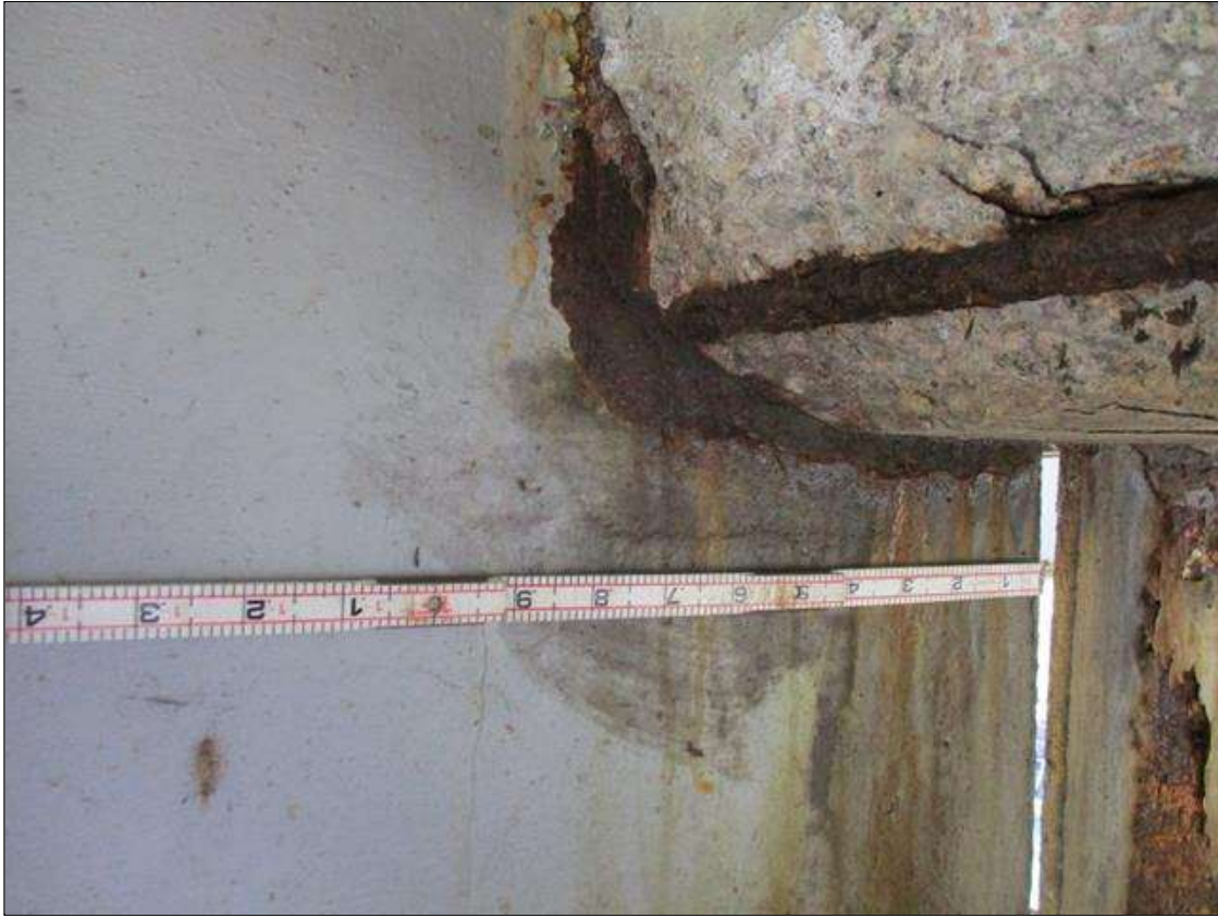
Span 7 Beam 2: [PROMPT ACTION REQUEST] BEAM END AT BENT 6, THERE IS AN APPROXIMATELY 1" WIDE BAND OF CORROSION THAT WRAPS THE REINFORCED CONCRETE DIAPHRAGM, APPROXIMATELY 3/16" SECTION LOSS [AVERAGE 1/4" REMAINS] FOR APPROXIMATELY 10" LONG.
