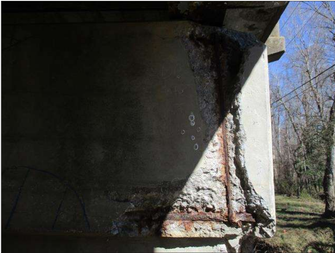
Bent 6 Cap 1: [PROMPT ACTION REQUEST] SOUTH FACE, RIGHT END, SPALLING WITH EXPOSED REBAR [APPROXIMATELY 2' LONG X FULL HEIGHT X UP TO 7" BACK X 3" DEEP]; SURFACE CORROSION AND PITTING TO 1/16" ON THE REBAR
