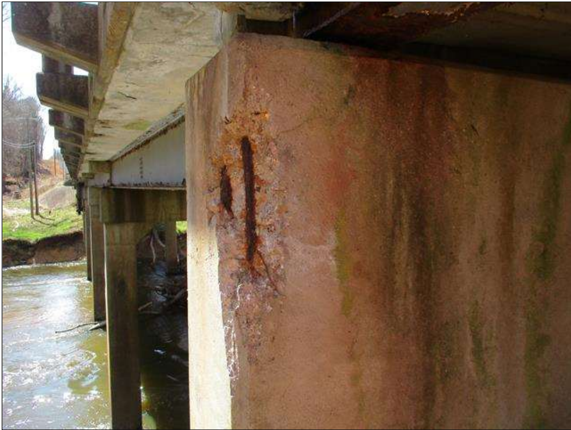
Bent 8 Cap 1: 18" X 7" X 3" DEEP SPALL WITH EXPOSED REBAR ON NORTHEAST CORNER
