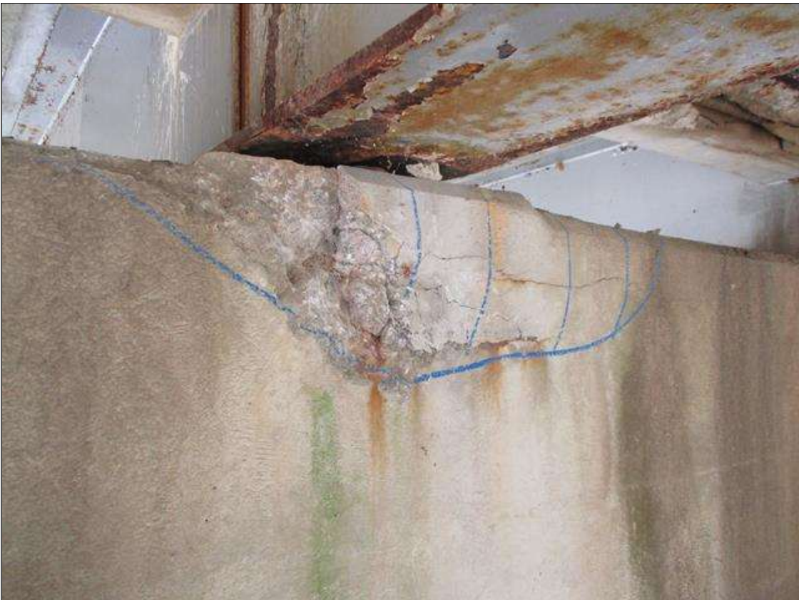
Bent 7 Cap 1: NORTH FACE AT BEAM 3, APPROXIMATELY 2 SQUARE FEET OF SPALLING AND MAP CRACKING TO 1/32" WIDE WITH ASSOCIATED DELAMINATION
