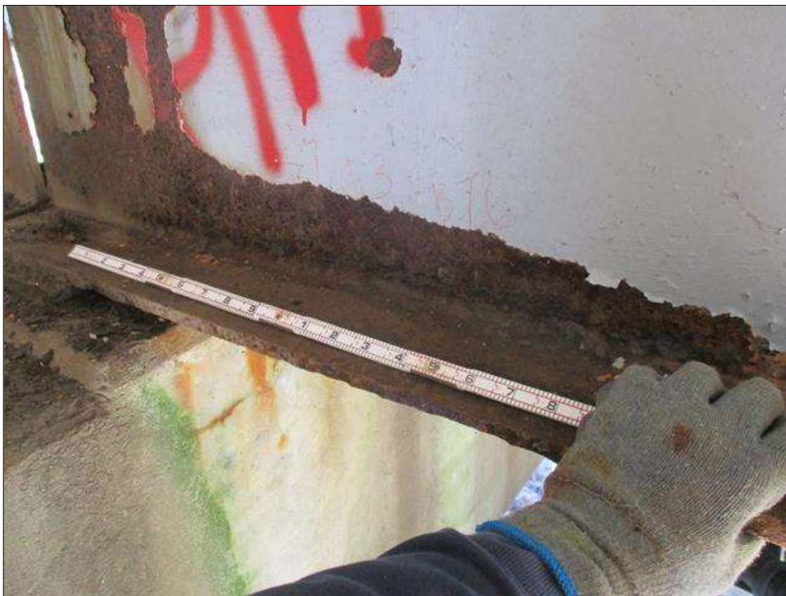
Span 7 Beam 3: [PROMPT ACTION REQUEST] 8" OUT FROM THE BEAM END AT BENT 6, IN THE LOWER 2" OF THE WEB, CORROSION WITH APPROXIMATELY 3/16" SECTION LOSS [AVERAGE 1/4" REMAINS] FOR 24" LONG.
