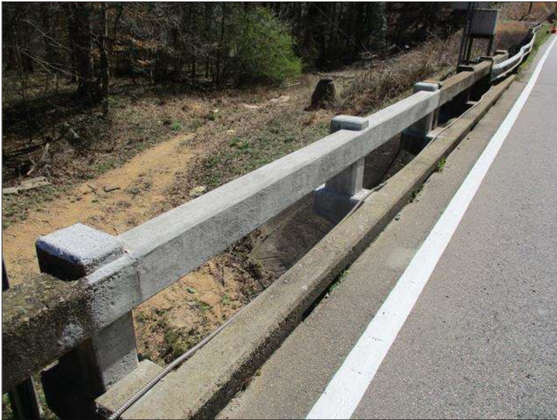
Span 2 Right Bridge Rail: APPROXIMATELY 12' OF SOUND PATCHING
