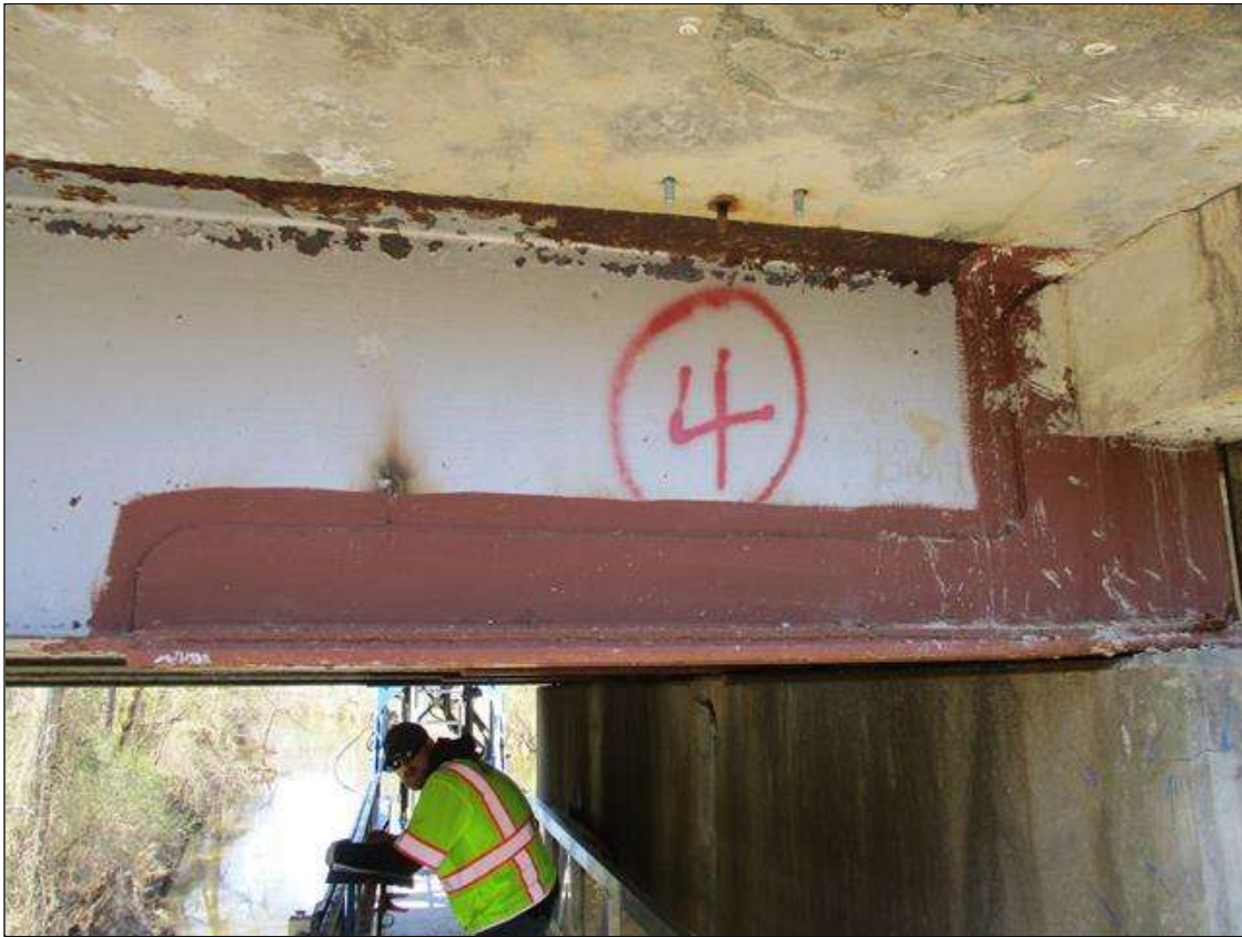
Span 5 Beam 4: [NEW REPAIR] BEAM END AT BENT 5, PLATES HAVE BEEN WELDED TO BOTH SIDES OF THE WEB [6' LONG X UP TO FULL HEIGHT] AND ON THE UPPER AND LOWER SIDES OF THE LOWER FLANGE [6' LONG X 1' WIDE] IN THE AREAS OF PAST SECTION LOSS.
