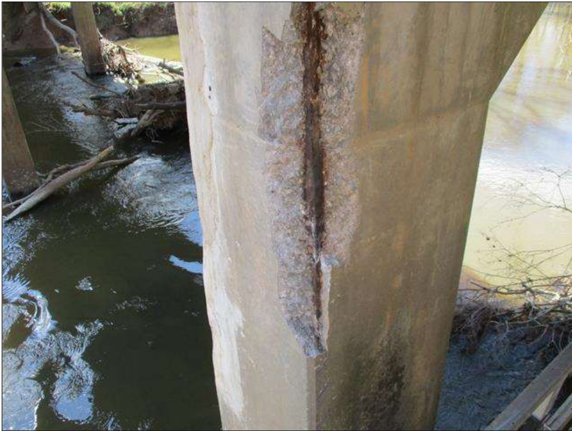
Bent 7 Pile 2: [PROMPT ACTION REQUEST] NORTHEAST CORNER, SPALLING WITH EXPOSED REBAR UP TO 2" DEEP, VERTICAL CRACKING TO 1/8" WIDE AND ASSOCIATED DELAMINATION [TOTAL AREA APPROXIMATELY 8' LONG X 1' WIDE]
