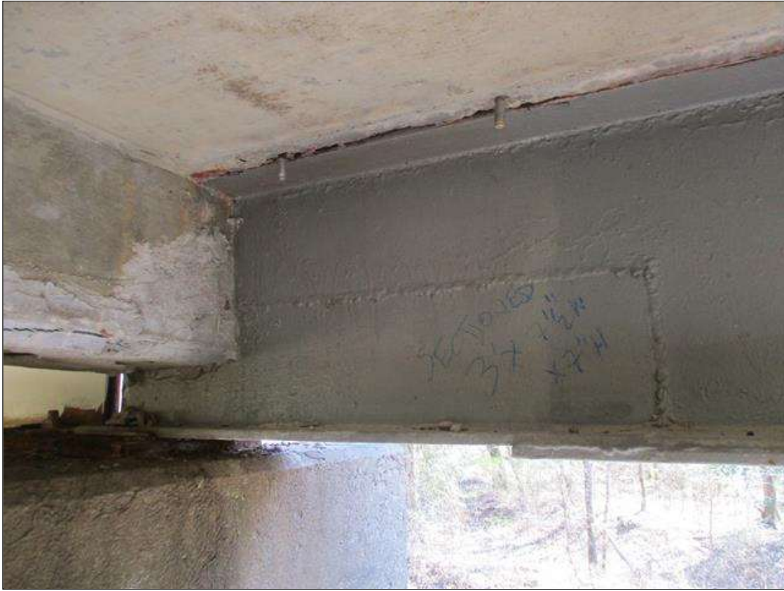
Span 1 Beam 6: [NEW REPAIR] BEAM END AT BENT 2 HAS BEEN SECTIONED, APPROXIMATELY 3' LONG X 7.5" WIDE X UP TO 7" HIGH
