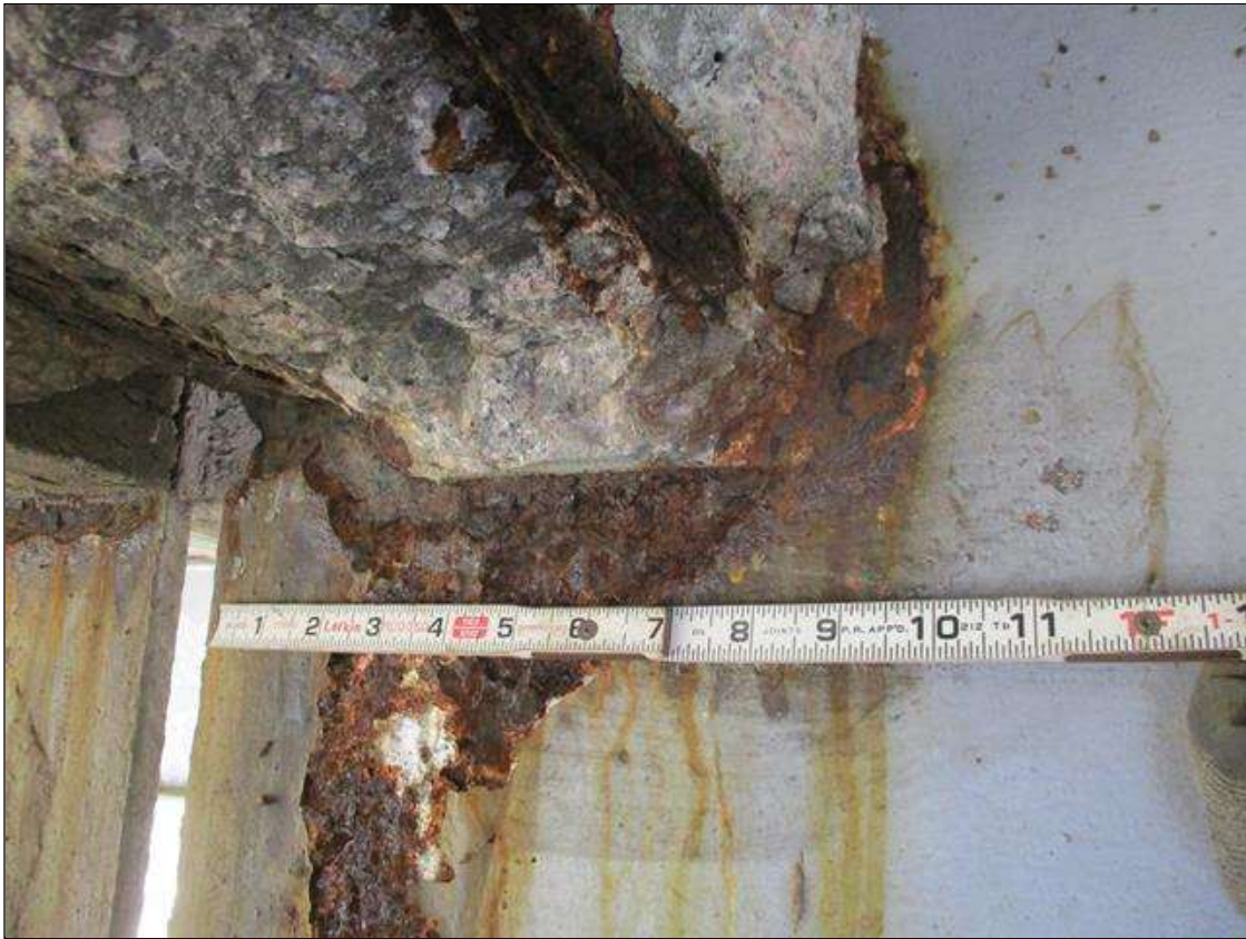
Span 5 Beam 2: [PROMPT ACTION REQUEST] BEAM END AT BENT 5, THERE IS AN APPROXIMATELY 1" WIDE BAND OF CORROSION THAT WRAPS THE REINFORCED CONCRETE DIAPHRAGM, APPROXIMATELY 1/4" SECTION LOSS [AVERAGE 3/16" REMAINS] FOR APPROXIMATELY 10" LONG.
