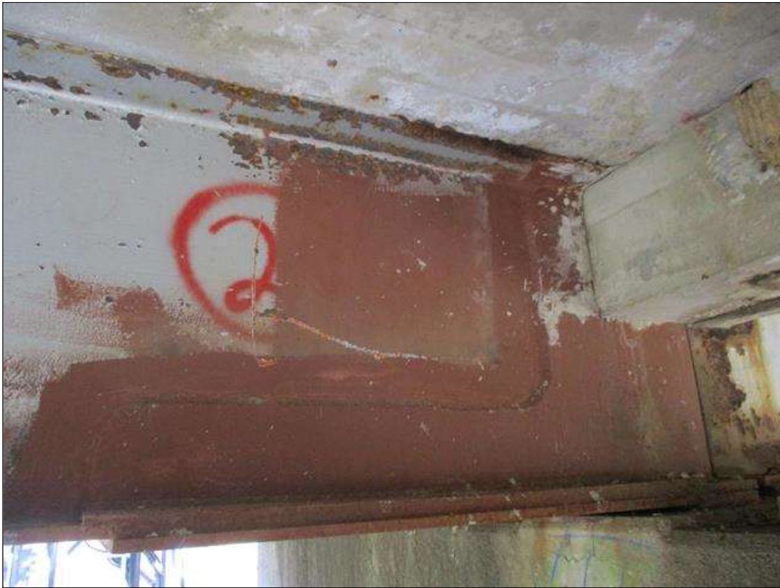
Span 5 Beam 2: [NEW REPAIR] BEAM END AT BENT 5, PLATES HAVE BEEN WELDED TO BOTH SIDES OF THE WEB [4' LONG X UP TO FULL HEIGHT] AND ON THE UPPER AND LOWER SIDES OF THE LOWER FLANGE [4' LONG X 1' WIDE] IN THE AREAS OF PAST SECTION LOSS.
