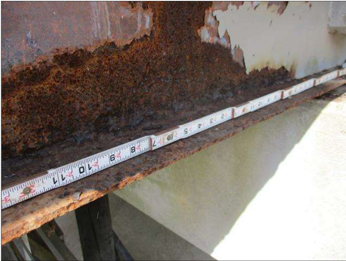
Span 9 Beam 6: [PROMPT ACTION REQUEST] BEAM END AT BENT 9, LOWER RIGHT FLANGE, CORROSION WITH APPROXIMATELY 1/4" SECTION LOSS [AVERAGE 3/16" REMAINS] FOR APPROXIMATELY 3' LONG, THEN AT 4' OUT, CORROSION WITH UP TO 3/8" SECTION LOSS [AVERAGE 1/16" REMAINS] WITH KNIFE EDGING AND CORROSION HOLES FOR APPROXIMATELY 3' LONG.
