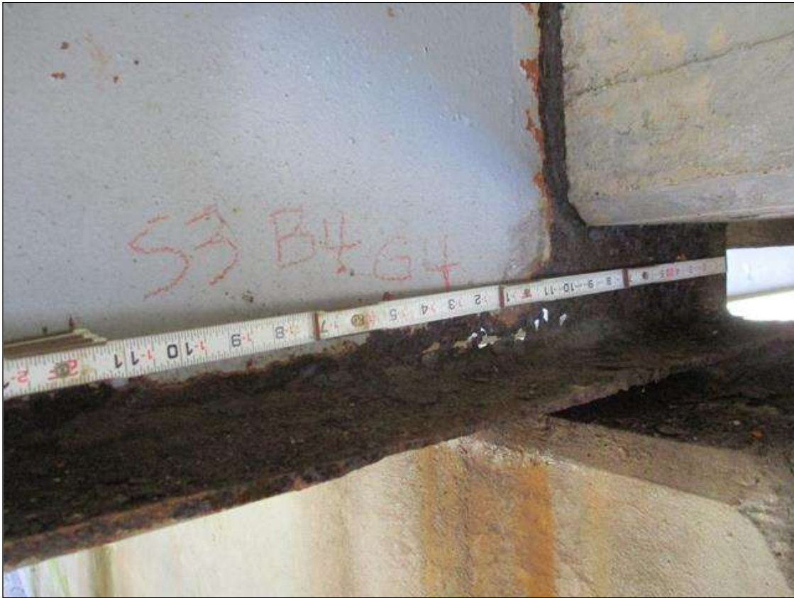
Span 3 Beam 4: [PROMPT ACTION REQUEST] APPROXIMATELY 6" OUT FROM THE BEAM END AT BENT 4, IN THE LOWER 2" OF THE WEB, CORROSION WITH APPROXIMATELY 1/8" SECTION LOSS [AVERAGE 3/16" REMAINS] FOR APPROXIMATELY 3" LONG, THEN 100% SECTION LOSS FOR APPROXIMATELY 6" LONG, THEN APPROXIMATELY 3/16" SECTION LOSS [AVERAGE 1/8" REMAINS] FOR APPROXIMATELY 12" LONG
