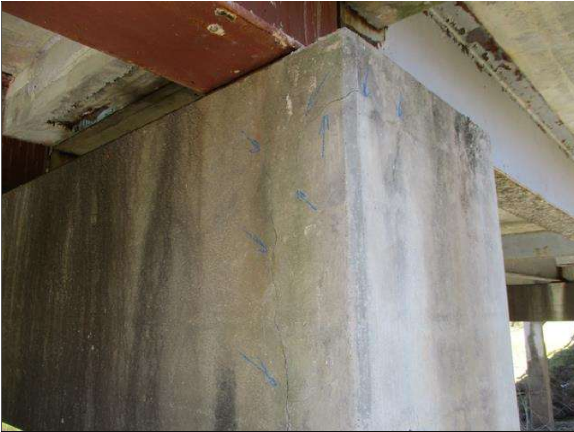
Bent 5 Cap 1: SOUTH FACE, RIGHT END, FULL HEIGHT MAP CRACKING TO 1/16" WIDE, EXTENDS BACK INTO THE EAST FACE UP TO 1'
