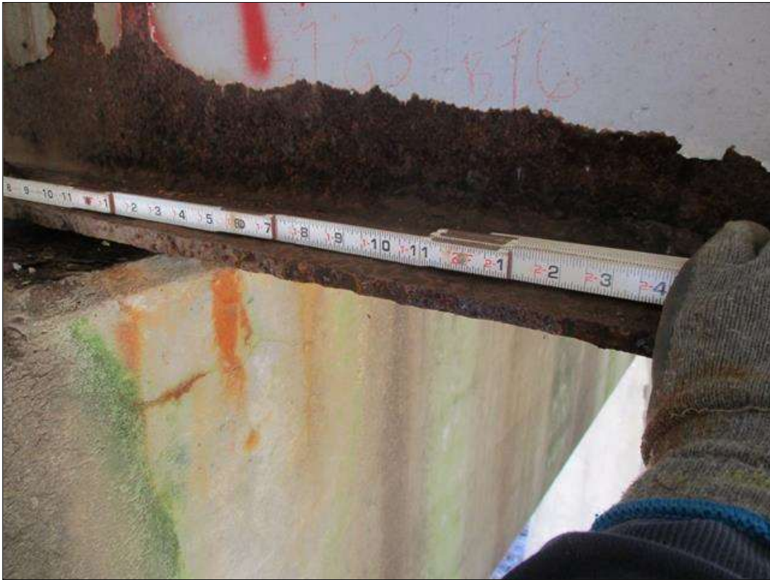
Span 7 Beam 3: [PROMPT ACTION REQUEST] BEAM END AT BENT 6, LOWER RIGHT FLANGE, CORROSION WITH APPROXIMATELY 5/16" SECTION LOSS [AVERAGE 5/16" REMAINS] FOR APPROXIMATELY 24" LONG
