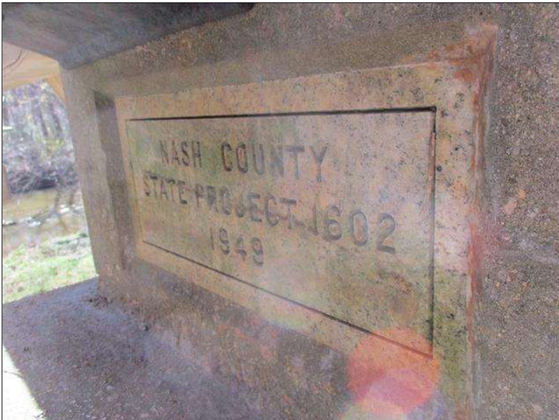
NORTHWEST CORNER, DATA PLATE
