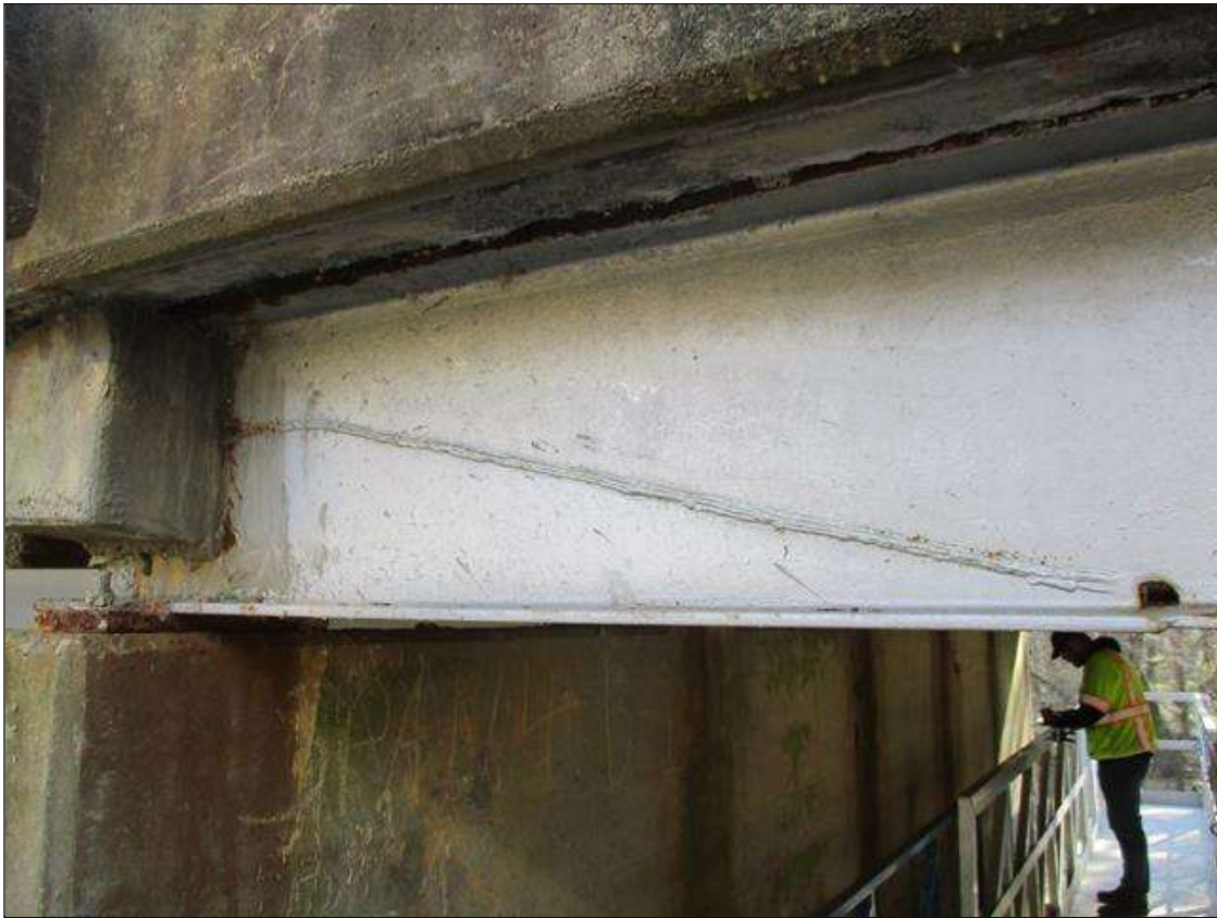
Span 4 Beam 1: [NEW REPAIR] BEAM END AT BENT 4 HAS BEEN SECTIONED, APPROXIMATELY 4.5' LONG X 7.5" WIDE X UP TO 9" HIGH
