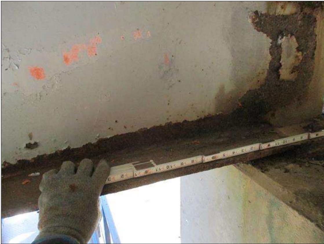
Span 5 Beam 1: [PROMPT ACTION REQUEST] 8" OUT FROM THE BEAM END AT BENT 5, IN THE LOWER 2" OF THE WEB, CORROSION WITH APPROXIMATELY 3/16" SECTION LOSS [AVERAGE 1/4" REMAINS] FOR 18" LONG.
