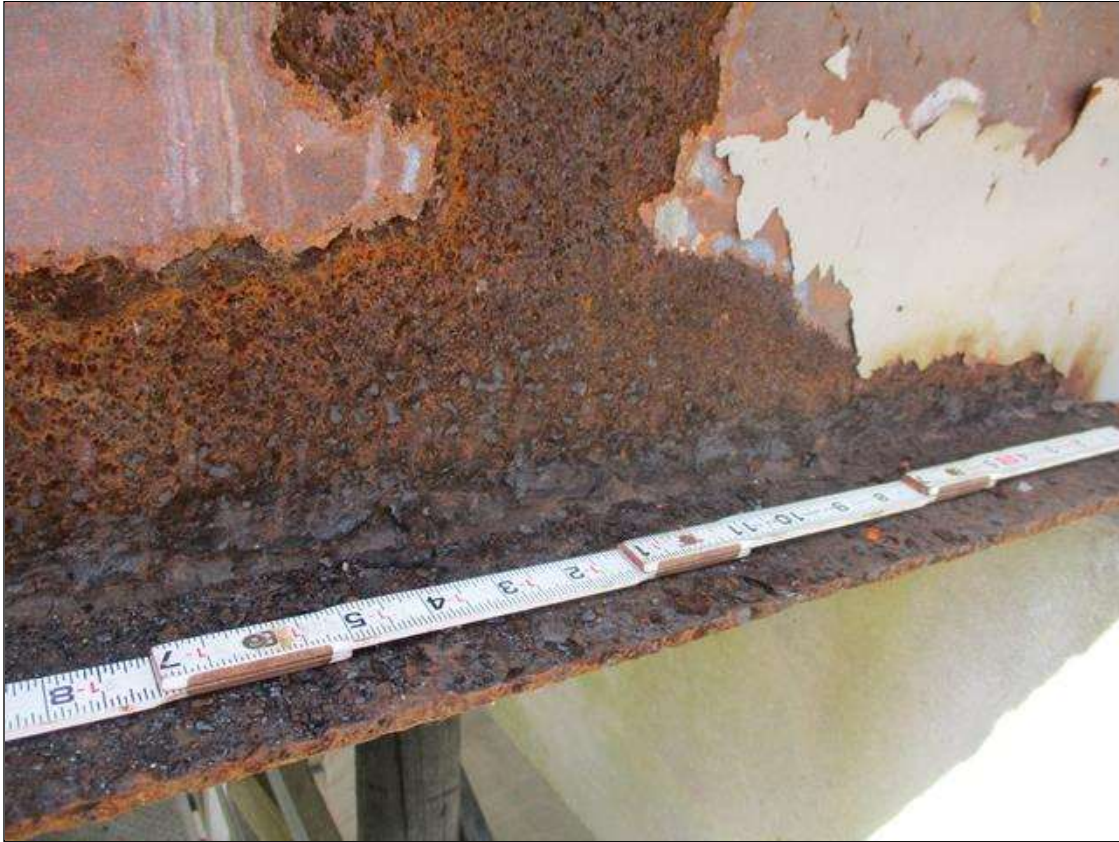
Span 9 Beam 6: [PROMPT ACTION REQUEST] APPROXIMATELY 5.5' OUT FROM THE BEAM END AT BENT 9, WEB, FULL HEIGHT, CORROSION WITH APPROXIMATELY 5/16" SECTION LOSS [AVERAGE 1/8" REMAINS] FOR 3" LONG. APPROXIMATELY 2' OUT FROM THE BEAM END AT BENT 9, WEB, LOWER AND UPPER 1", CORROSION WITH APPROXIMATELY 5/16" SECTION LOSS [AVERAGE 1/8" REMAINS] FOR 12" LONG.
