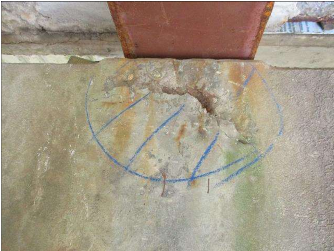
Bent 5 Cap 1: SOUTH FACE AT BEAM 3, TOP, APPROXIMATELY 1.5 SQUARE FEET MAP CRACKING TO 1/16" WIDE WITH ASSOCIATED DELAMINATION
