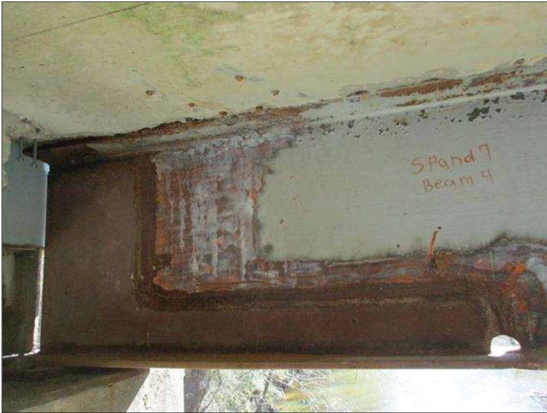
Span 7 Beam 4: [NEW REPAIR] BEAM END AT BENT 7, BEAM END HAS BEEN SECTIONED [4.5' LONG X UP TO 26" HIGH]
