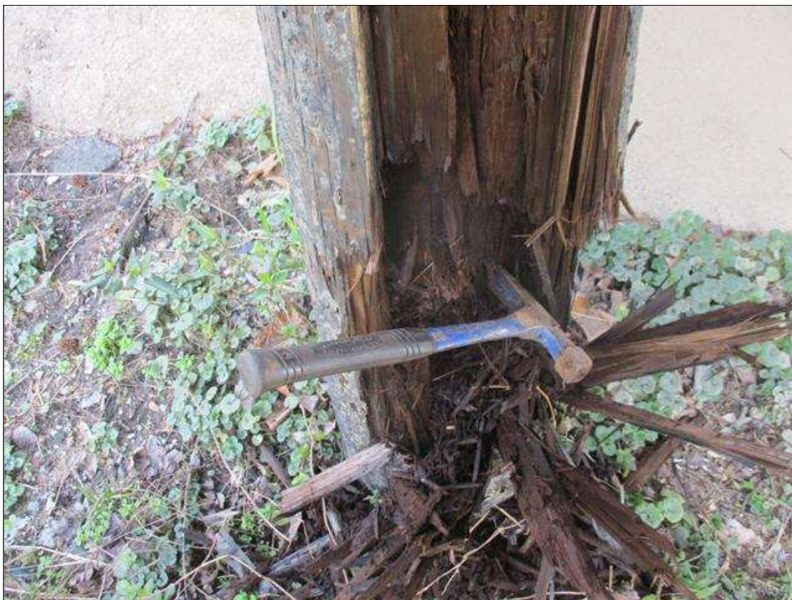
Bent 9 Pile 1: [PROMPT ACTION REQUEST] AT THE GROUNDLINE, DECAY AND SECTION LOSS WITH APPROXIMATELY 4" CORE REMAINING FOR APPROXIMATELY 4' HIGH
