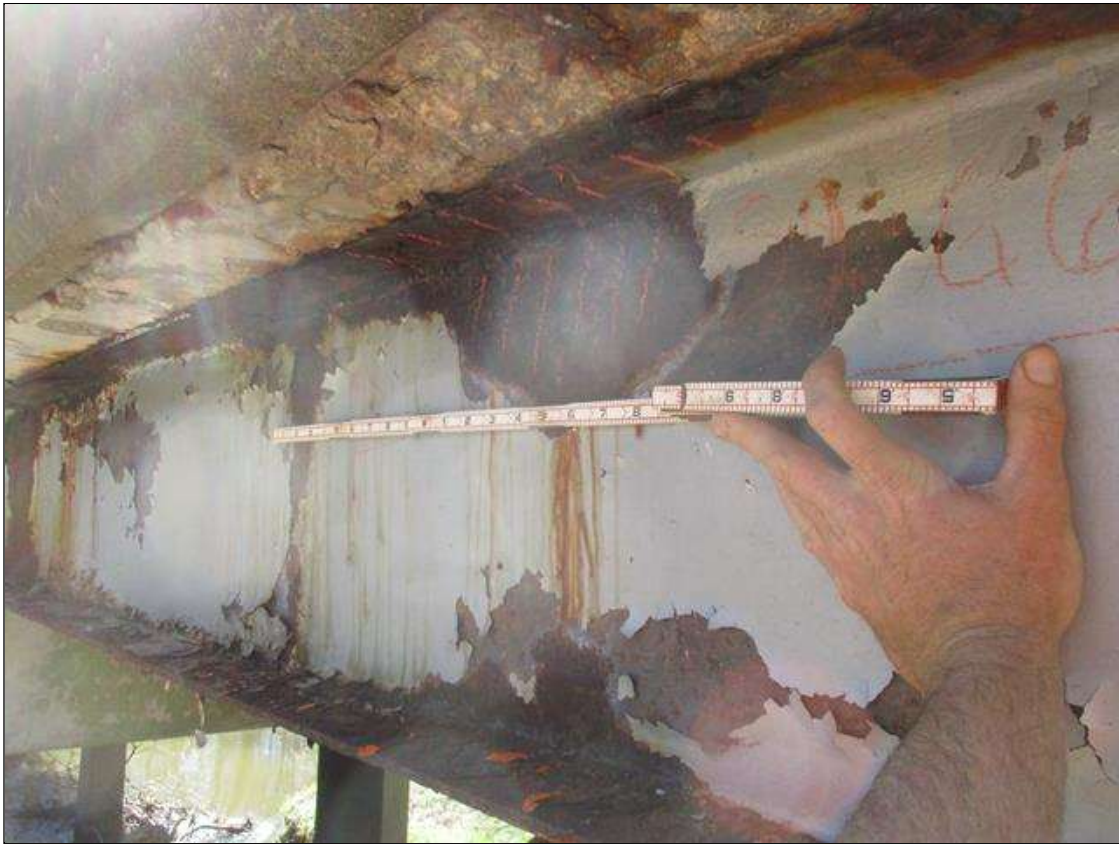
Span 9 Beam 6: [PROMPT ACTION REQUEST] 5/16" SECTION LOSS (1/8" REMAINING) ON TOP RIGHT FLANGE FOR HALF FLANGE WIDTH FOR 5' STARTING 10' FROM BENT 9 IN SPAN 10 WITH SCATTERED SECTION LOSS TO 1/8" [AVERAGE 3/16" REMAINING] IN THE UPPER AND LOWER 3" OF THE WEB AT THIS LOCATION
