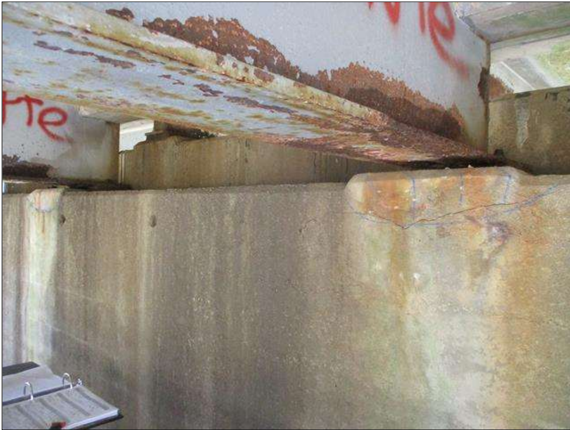
Bent 4 Cap 1: NORTH FACE AT BEAMS 2 & 3, (2) AREAS OF MAP CRACKING TO 1/8" WIDE WITH ASSOCIATED DELAMINATION
