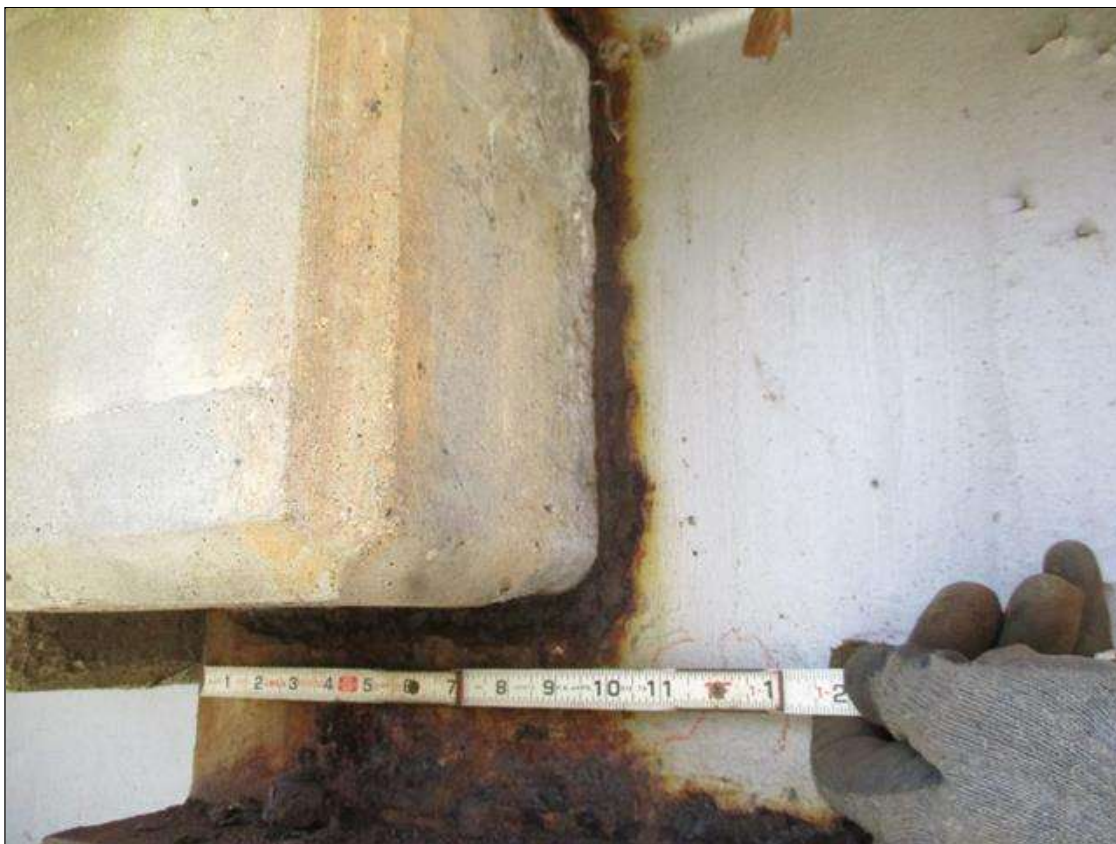
Span 9 Beam 6: [PROMPT ACTION REQUEST] BEAM END AT BENT 8, THERE IS AN APPROXIMATELY 1" WIDE BAND OF CORROSION THAT WRAPS THE REINFORCED CONCRETE DIAPHRAGM, APPROXIMATELY 3/16" SECTION LOSS [AVERAGE 3/16" REMAINS] FOR APPROXIMATELY 10" LONG.
