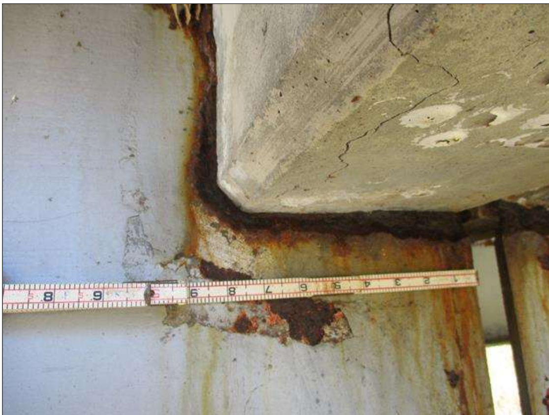
Span 5 Beam 4: [PROMPT ACTION REQUEST] BEAM END AT BENT 5, THERE IS AN APPROXIMATELY 1" WIDE BAND OF CORROSION THAT WRAPS THE REINFORCED CONCRETE DIAPHRAGM, APPROXIMATELY 1/4" SECTION LOSS [AVERAGE 3/16" REMAINS] FOR APPROXIMATELY 10" LONG.
