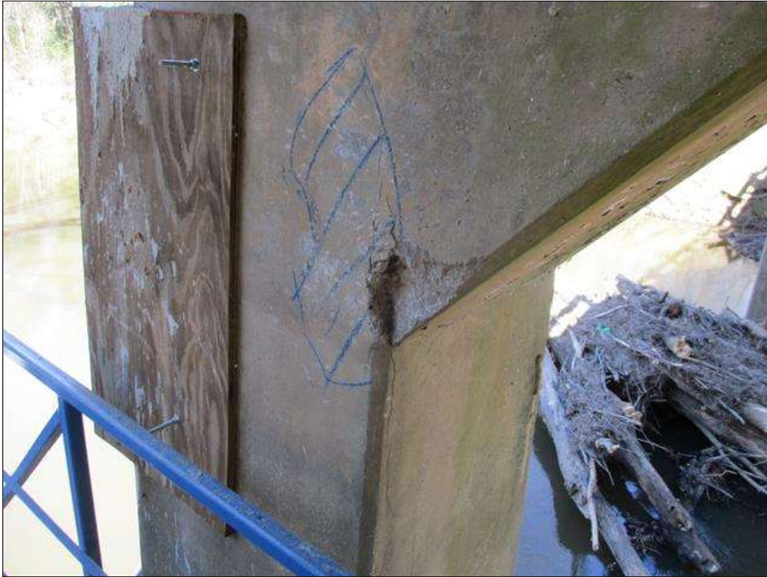
Bent 5 Pile 1: AT THE HAUNCH, APPROXIMATELY 2 SQUARE FEET MAP CRACKING TO 1/16" WIDE WITH ASSOCIATED DELAMINATION AND SPALLING TO 2" DEEP
