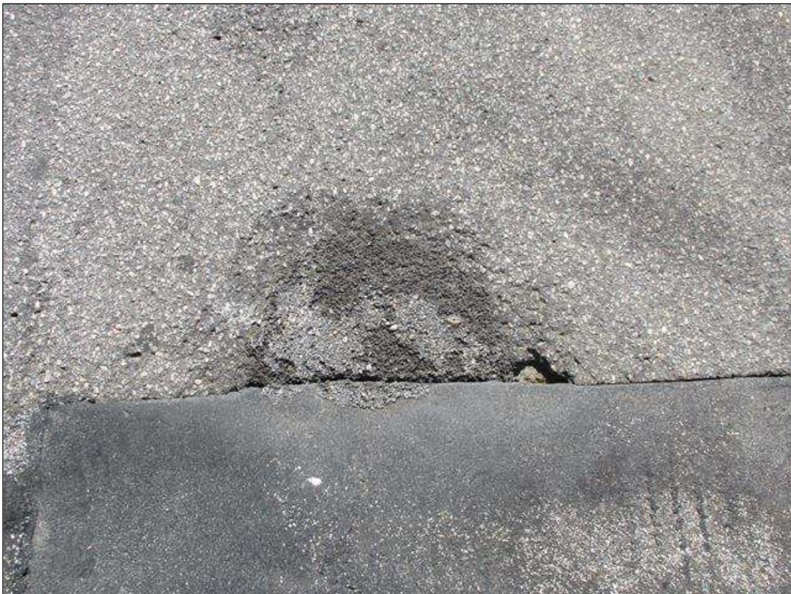
Span 2 Wearing Surface: LEFT LANE AT BENT 2, APPROXIMATELY 2 SQUARE FEET UNSOUND PATCHING [COLD PATCH]
