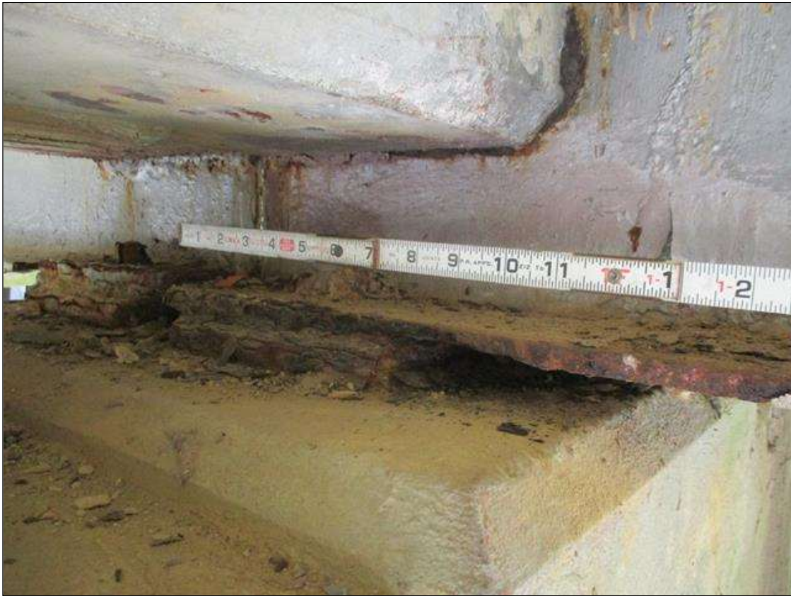
Span 3 Beam 4: [PROMPT ACTION REQUEST] APPROXIMATELY 6" OUT FROM THE BEAM END AT BENT 2, LOWER RIGHT FLANGE, CORROSION WITH APPROXIMATELY 1/8" SECTION LOSS [AVERAGE 1/4" REMAINS] FOR APPROXIMATELY 4" LONG
