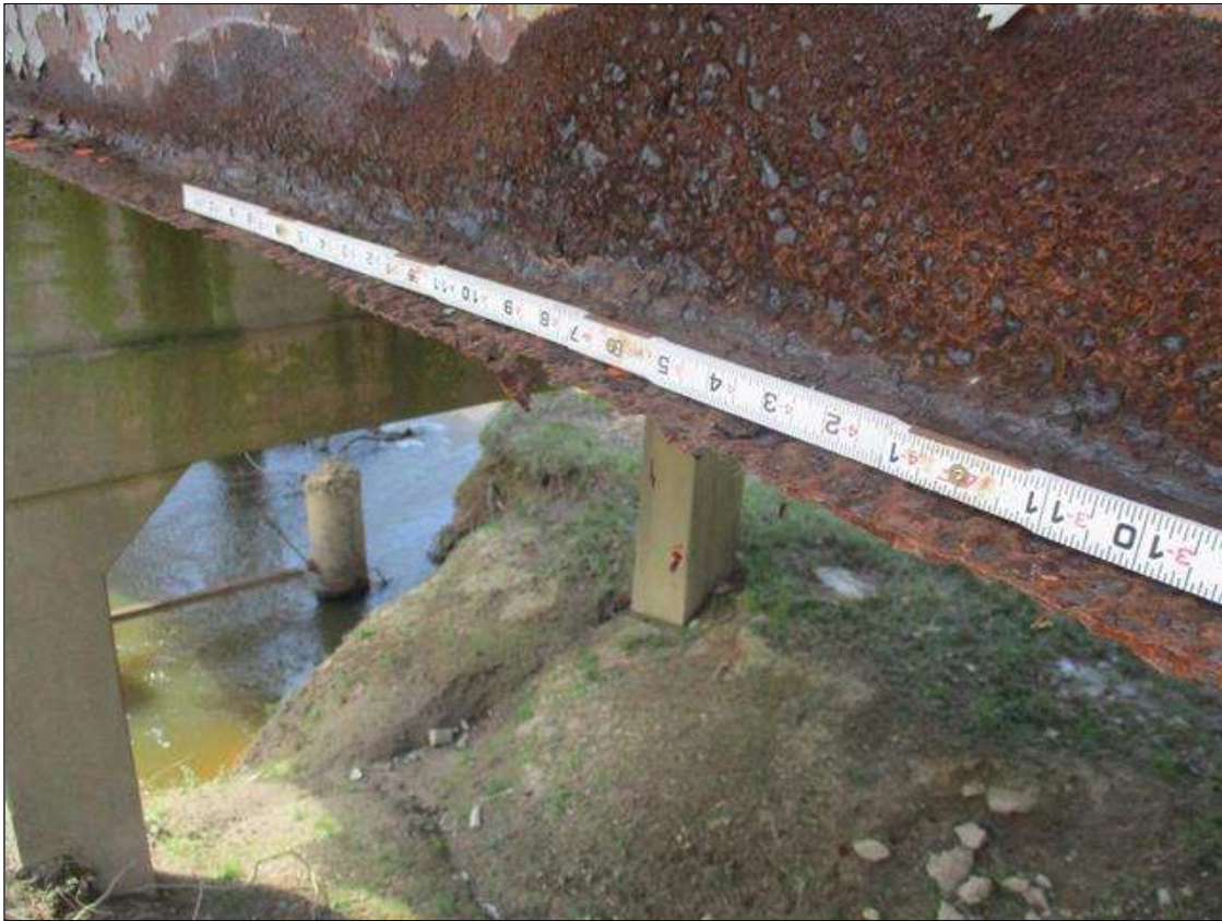
Span 9 Beam 6: [PROMPT ACTION REQUEST] BEAM END AT BENT 9, LOWER RIGHT FLANGE, CORROSION WITH APPROXIMATELY 1/4" SECTION LOSS [AVERAGE 3/16" REMAINS] FOR APPROXIMATELY 3' LONG, THEN AT 4' OUT, CORROSION WITH UP TO 3/8" SECTION LOSS [AVERAGE 1/16" REMAINS] WITH KNIFE EDGING AND CORROSION HOLES FOR APPROXIMATELY 3' LONG.
