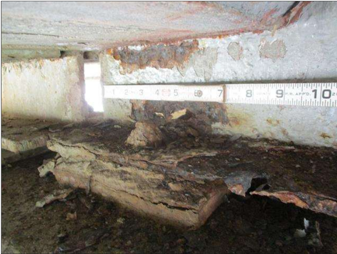
Span 1 Beam 3: [PROMPT ACTION REQUEST] APPROXIMATELY 2" OUT FROM THE BEAM END AT BENT 2, IN THE LOWER 1" OF THE WEB, CORROSION WITH 100% SECTION LOSS FOR APPROXIMATELY 4" LONG.
