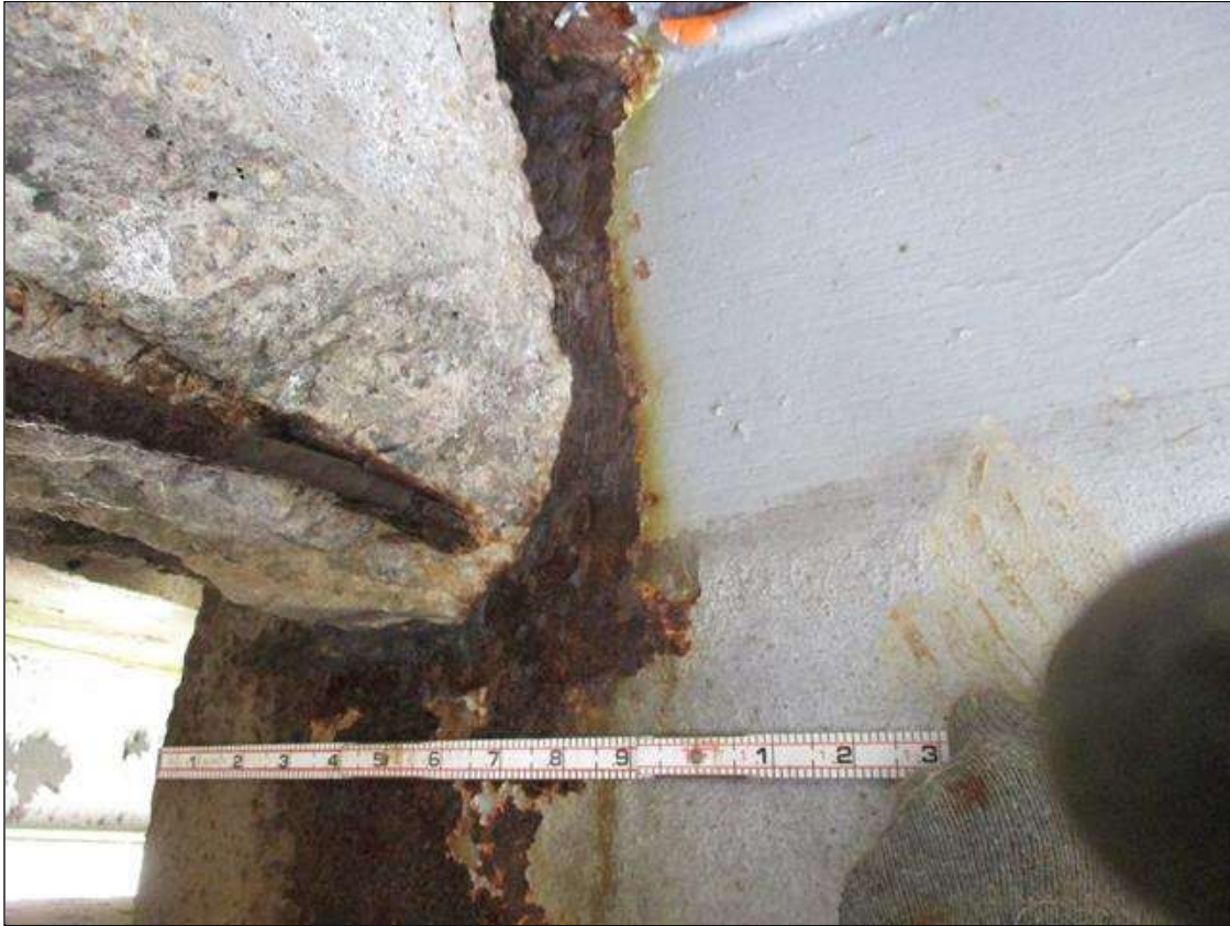
Span 8 Beam 3: [PROMPT ACTION REQUEST] BEAM END AT BENT 8, THERE IS AN APPROXIMATELY 2" WIDE BAND OF CORROSION THAT WRAPS THE REINFORCED CONCRETE DIAPHRAGM, APPROXIMATELY 1/4" SECTION LOSS [AVERAGE 3/16" REMAINS] FOR APPROXIMATELY 10" LONG.
