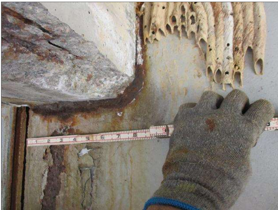
Span 8 Beam 3: [PROMPT ACTION REQUEST] BEAM END AT BENT 7, THERE IS AN APPROXIMATELY 1" WIDE BAND OF CORROSION THAT WRAPS THE REINFORCED CONCRETE DIAPHRAGM, APPROXIMATELY 1/4" SECTION LOSS [AVERAGE 3/16" REMAINS] FOR APPROXIMATELY 10" LONG.
