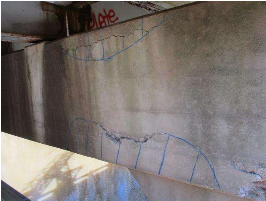
Bent 6 Cap 1: SOUTH FACE AT BAY 3, UPPER AND LOWER 12" OF THE CAP FACE, MAP CRACKING TO 1/8" WIDE WITH APPROXIMATELY 6 SQUARE FEET OF ASSOCIATED DELAMINATION
