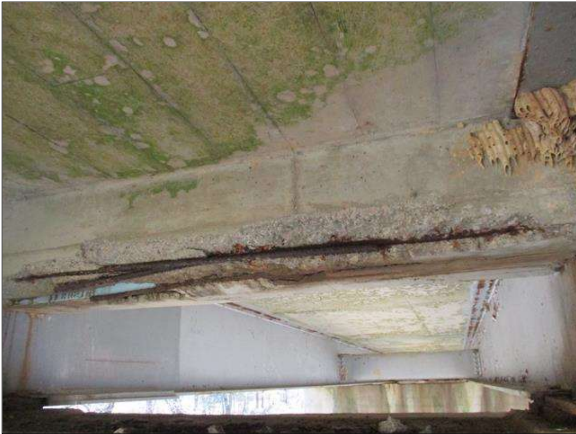
Span 8 Beam 2: [PROMPT ACTION REQUEST] BAY 2 AT BENT 7, REINFORCED CONCRETE DIAPHRAGM, SPALLING WITH EXPOSED REBAR [APPROXIMATELY 5' LONG X 10" WIDE X UP TO 3" DEEP]. THE REBAR IS DELAMINATED FROM THE CONCRETE AND HAS SURFACE CORROSION AND PITTING UP TO 1/16" DEEP.
