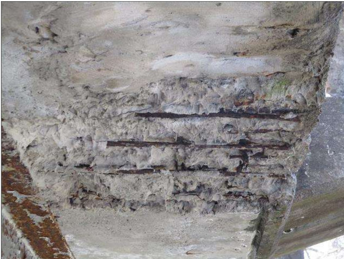
Span 5 Deck: [PROMPT ACTION REQUEST] 5' X 2' X 3" DEEP SPALLING WITH HEAVILY DECAYED REBAR [SECTION LOSS UP TO 100%] IN LEFT OVERHANG AT 7' FROM BENT 5
