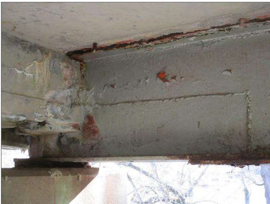
Span 4 Beam 6: [NEW REPAIR] BEAM END AT BENT 4 HAS BEEN SECTIONED, APPROXIMATELY 3' LONG X 7.5" WIDE X UP TO 7" HIGH
