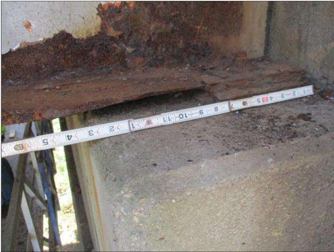
Span 8 Beam 4: [PROMPT ACTION REQUEST] BEAM END AT BENT 8, LOWER RIGHT FLANGE, CORROSION WITH APPROXIMATELY 3/8" SECTION LOSS [AVERAGE 1/4" REMAINS] FOR APPROXIMATELY 1' LONG.
