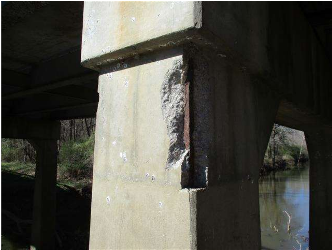
Bent 6 Pile 2: [PROMPT ACTION REQUEST] ON SOUTHEAST AND NORTHEAST CORNERS, SPALLING WITH EXPOSED REBAR [UP TO 2' LONG X 8" WIDE X 2" DEEP], NO MEASURABLE SECTION LOSS
