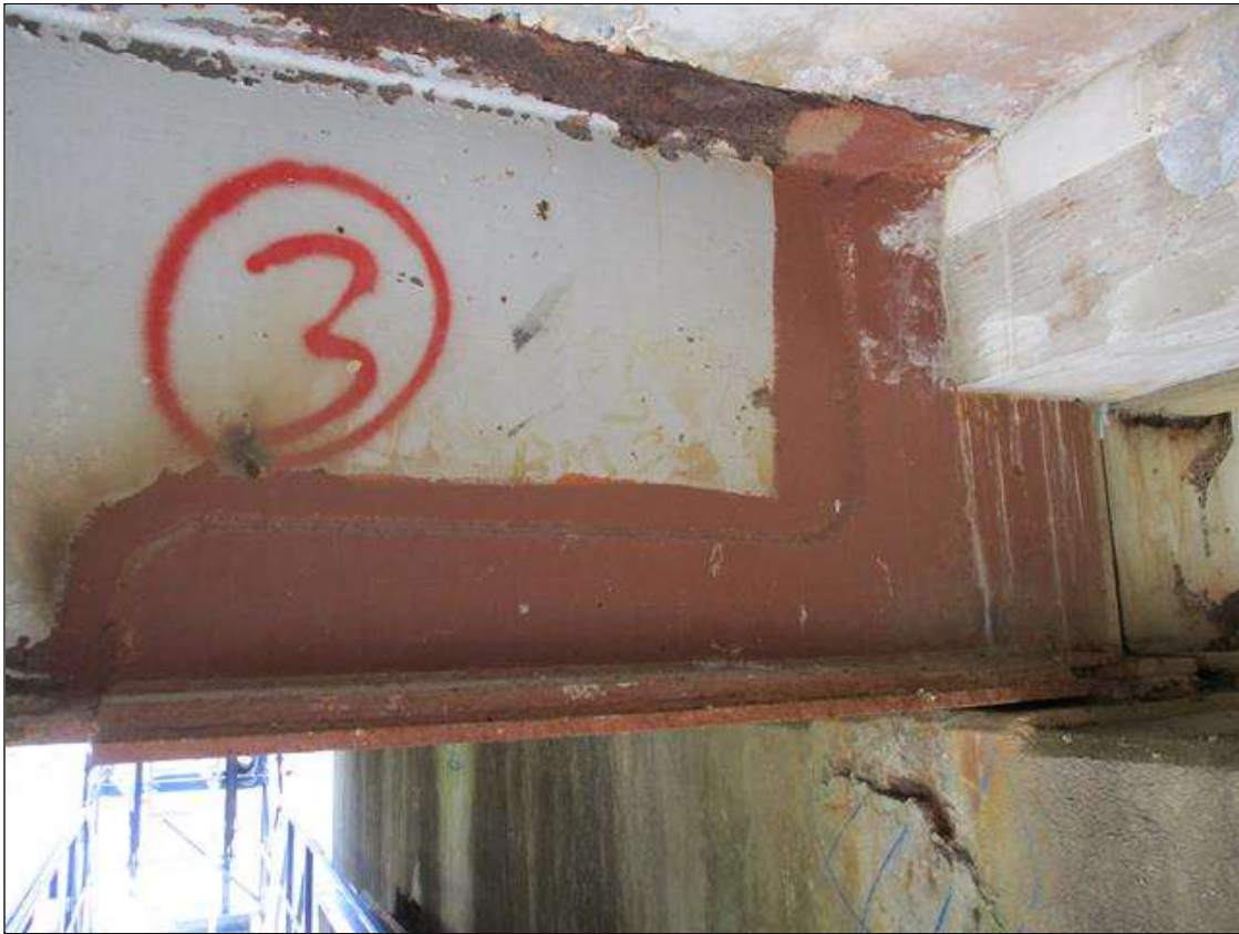
Span 5 Beam 3: [NEW REPAIR] BEAM END AT BENT 5, PLATES HAVE BEEN WELDED TO BOTH SIDES OF THE WEB [4' LONG X UP TO FULL HEIGHT] AND ON THE UPPER AND LOWER SIDES OF THE LOWER FLANGE [4' LONG X 1' WIDE] IN THE AREAS OF PAST SECTION LOSS.
