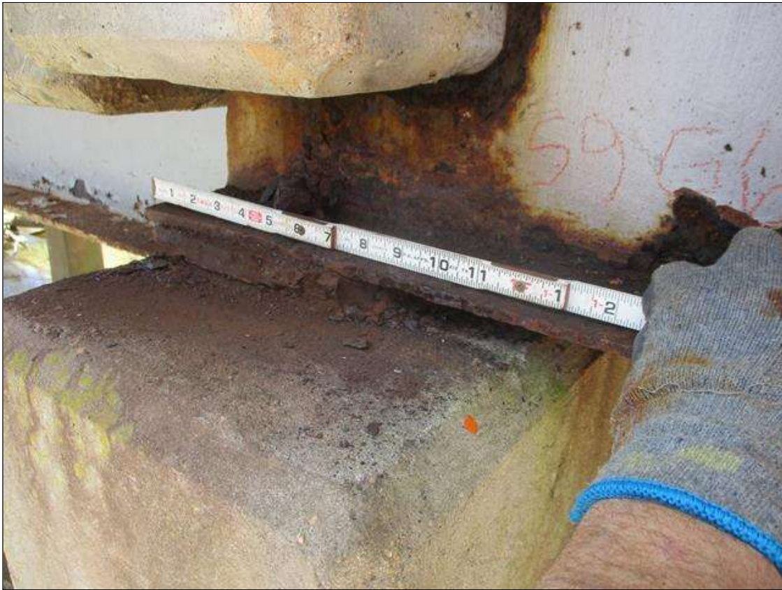
Span 9 Beam 6: [PROMPT ACTION REQUEST] APPROXIMATELY 8" OUT FROM THE BEAM END AT BENT 8, LOWER RIGHT FLANGE, CORROSION WITH APPROXIMATELY 3/16" SECTION LOSS [AVERAGE 1/4" REMAINS] FOR APPROXIMATELY 1' LONG.
