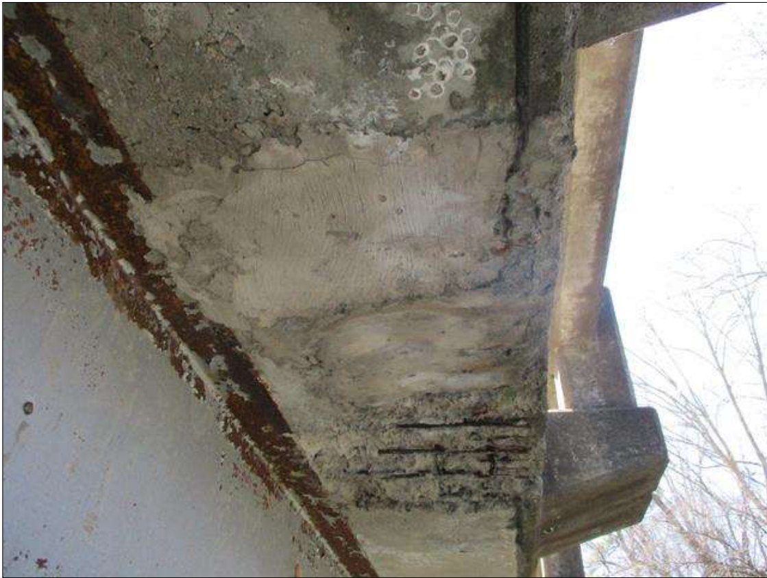
Span 5 Deck: [PROMPT ACTION REQUEST] 5' X 2' X 3" DEEP SPALLING WITH HEAVILY DECAYED REBAR [SECTION LOSS UP TO 100%] IN LEFT OVERHANG AT 7' FROM BENT 5
