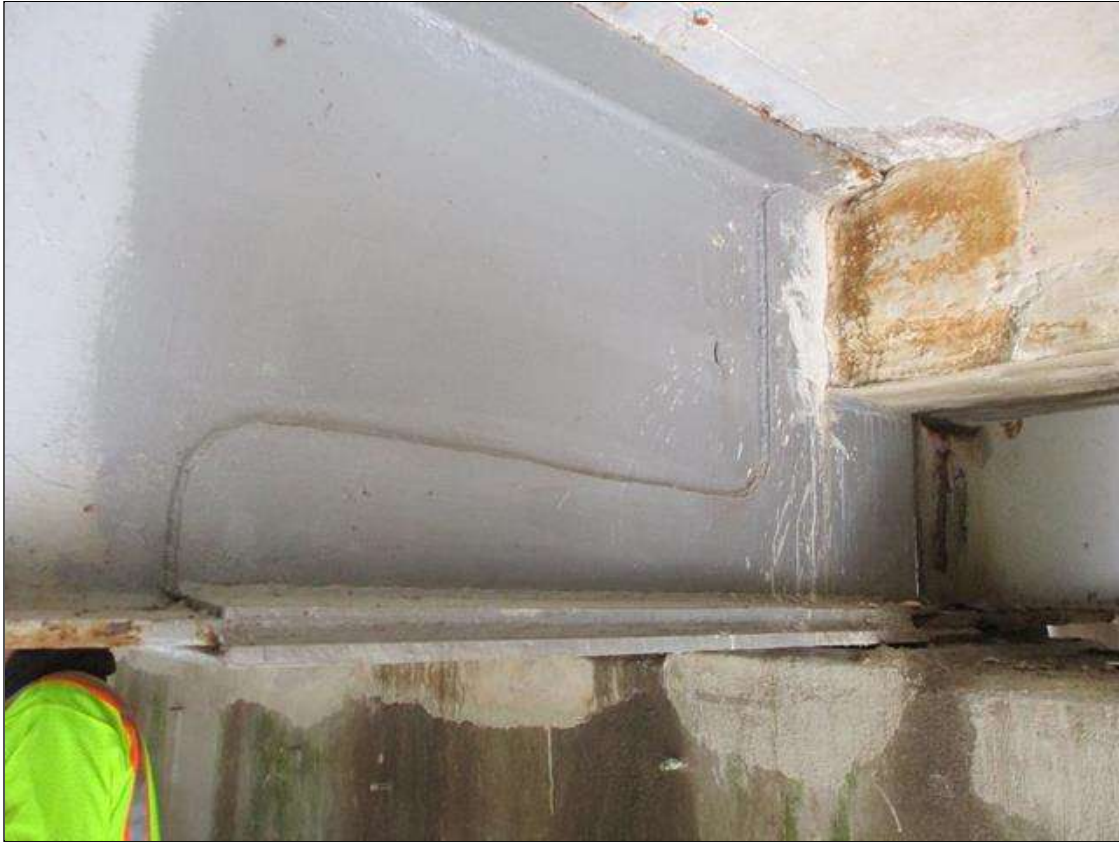
Span 7 Beam 3: [NEW REPAIR] BEAM END AT BENT 7, PLATES HAVE BEEN WELDED TO BOTH SIDES OF THE WEB [4' LONG X UP TO FULL HEIGHT] AND ON THE UPPER AND LOWER SIDES OF THE LOWER FLANGE [3.33' LONG X 11-3/4" WIDE] IN THE AREAS OF PAST SECTION LOSS.
