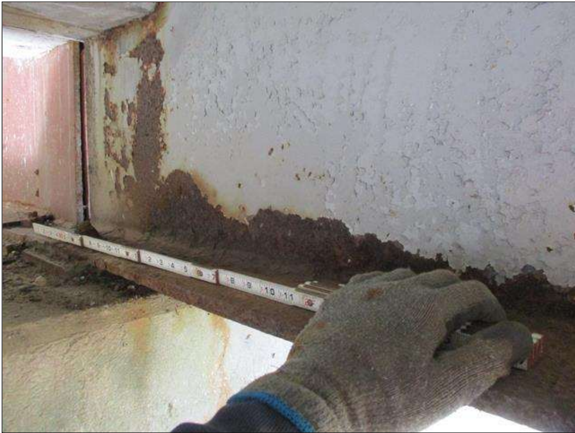
Span 6 Beam 1: [PROMPT ACTION REQUEST] BEAM END AT BENT 5, IN THE LOWER 2" OF THE WEB, CORROSION WITH APPROXIMATELY 1/8" SECTION LOSS [AVERAGE 5/16" REMAINS] FOR 24" LONG.
