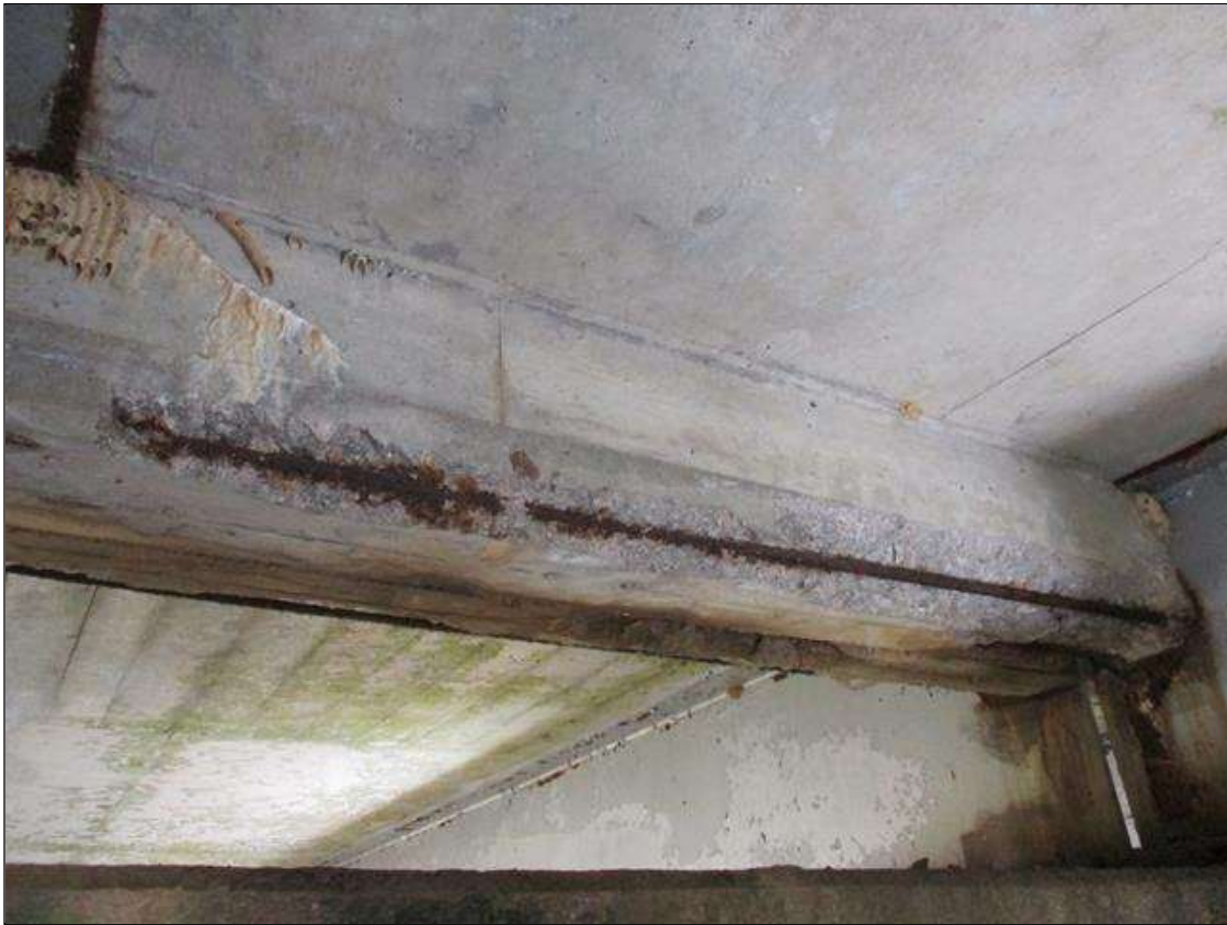
Span 5 Beam 1: [PROMPT ACTION REQUEST] BAY 1 AT BENT 5, REINFORCED CONCRETE DIAPHRAGM, SPALLING WITH EXPOSED REBAR [APPROXIMATELY 6' LONG X 8" WIDE X UP TO 2" DEEP] WITH DELAMINATED REBAR, WHICH HAS SURFACE CORROSION AND PITTING UP TO 1/8" DEEP
