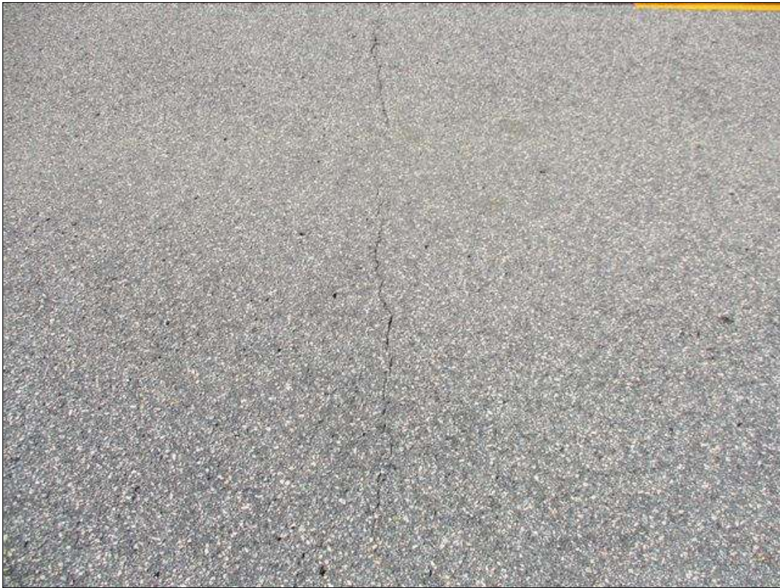
Span 5 Wearing Surface: SCATTERED LONGITUDINAL CRACKING TO 3/16" WIDE
