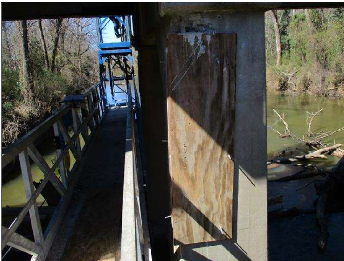
Bent 5 Pile 2: SOUND PATCHING --> [FORMERLY 4' X 10" X 9" DEEP SPALL WITH EXPOSED REBAR]
