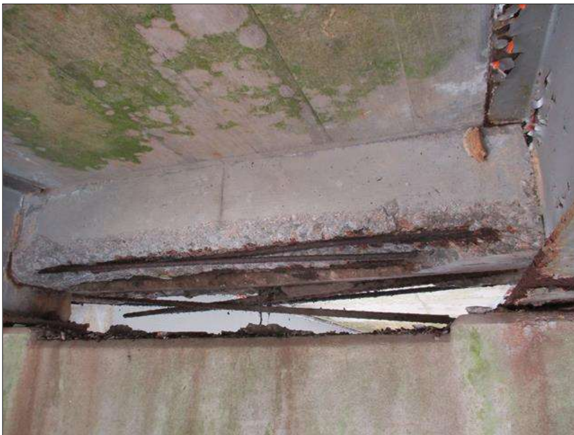
Span 9 Beam 3: [PROMPT ACTION REQUEST] BAY 3 AT BENT 8, REINFORCED CONCRETE DIAPHRAGM, SPALLING WITH EXPOSED REBAR [APPROXIMATELY 5' LONG X 9" WIDE X UP TO 3" DEEP]. THE REBAR IS DELAMINATED FROM THE CONCRETE AND HAS SURFACE CORROSION AND PITTING UP TO 1/16" DEEP.
