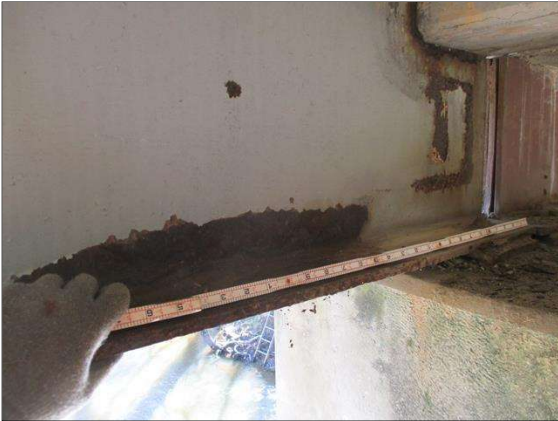
Span 6 Beam 4: [PROMPT ACTION REQUEST] 15" OUT FROM THE BEAM END AT BENT 5, IN THE LOWER 2" OF THE WEB, CORROSION WITH APPROXIMATELY 1/8" SECTION LOSS [AVERAGE 5/16" REMAINS] FOR 18" LONG.
