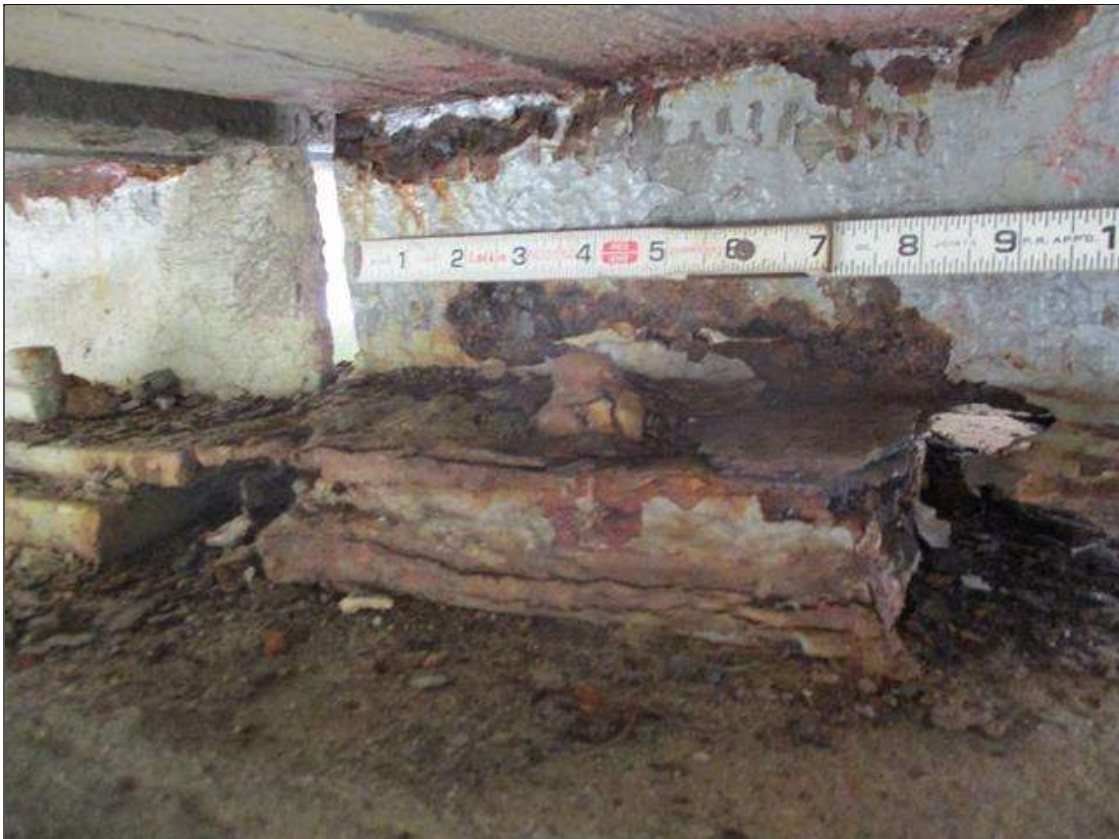
Span 1 Beam 5: [PROMPT ACTION REQUEST] APPROXIMATELY 2" OUT FROM THE BEAM END AT BENT 2, IN THE LOWER 1" OF THE WEB, CORROSION WITH 100% SECTION LOSS FOR APPROXIMATELY 5" LONG.
