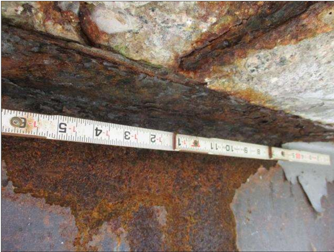
Span 9 Beam 6: [PROMPT ACTION REQUEST] BEAM END AT BENT 9, UPPER RIGHT FLANGE, CORROSION WITH APPROXIMATELY 1/4" SECTION LOSS [AVERAGE 3/16" REMAINS] FOR APPROXIMATELY 7' LONG.
