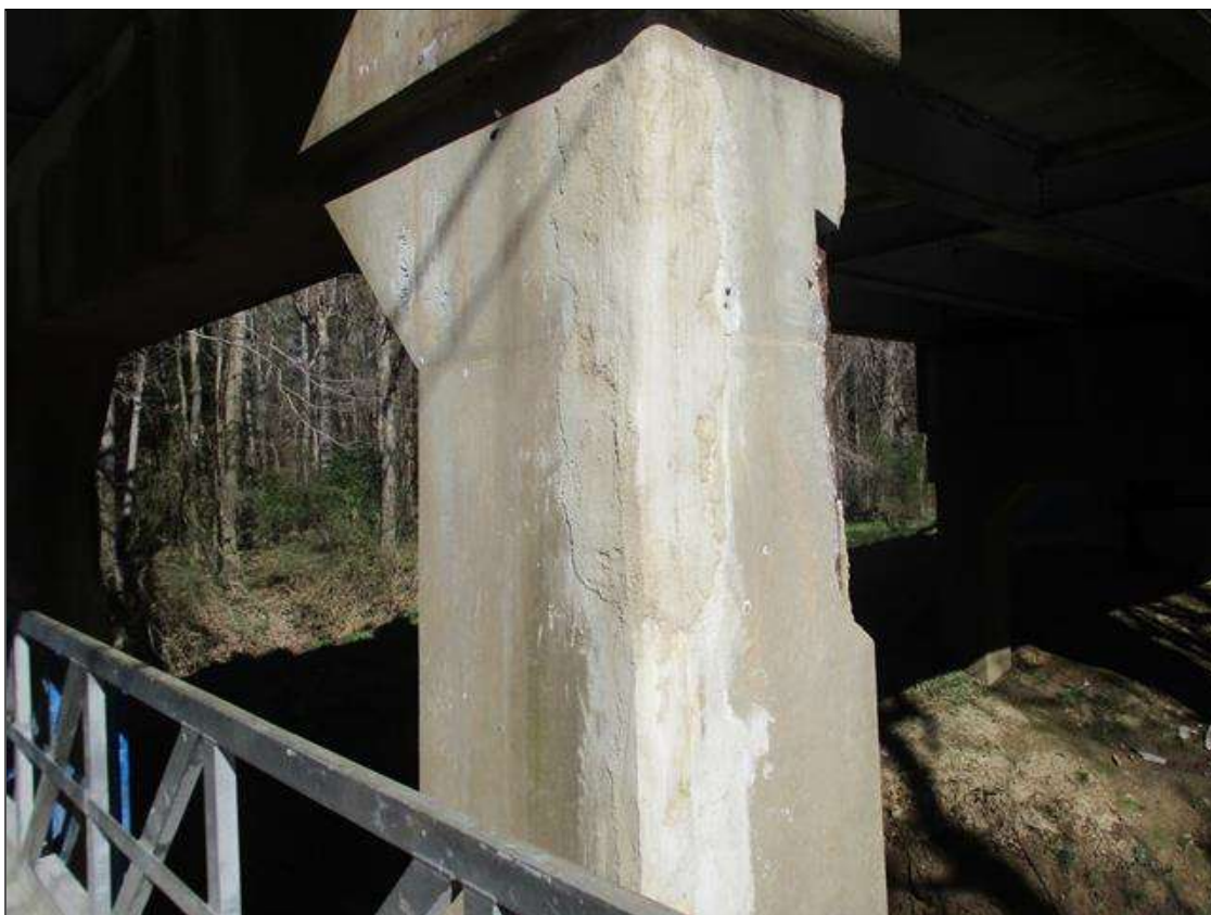
Bent 7 Pile 2: [NEW REPAIR] SOUND PATCHING --> FORMERLY 3.5' X 7" X 8" SPALL WITH EXPOSED REBAR ON SOUTHEAST CORNER
