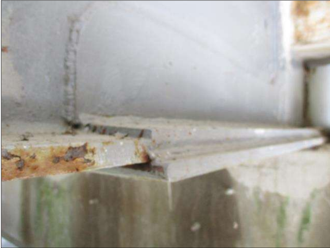
[NEW REPAIR] BEAM END AT BENT 7, PLATES HAVE BEEN WELDED TO BOTH SIDES OF THE WEB [4' LONG X UP TO FULL HEIGHT] AND ON THE UPPER AND LOWER SIDES OF THE LOWER FLANGE [3.33' LONG X 11-3/4" WIDE] IN THE AREAS OF PAST SECTION LOSS. [TYPICAL FOR THIS REPAIR]
