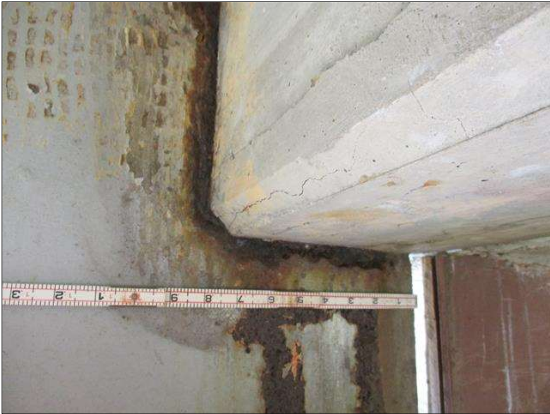
Span 6 Beam 4: [PROMPT ACTION REQUEST] BEAM END AT BENT 5, THERE IS AN APPROXIMATELY 1" WIDE BAND OF CORROSION THAT WRAPS THE REINFORCED CONCRETE DIAPHRAGM, APPROXIMATELY 1/8" SECTION LOSS [AVERAGE 5/16" REMAINS] FOR APPROXIMATELY 10" LONG.
