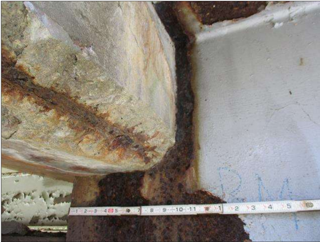
Span 8 Beam 1: [PROMPT ACTION REQUEST] BEAM END AT BENT 8, THERE IS AN APPROXIMATELY 1" WIDE BAND OF CORROSION THAT WRAPS THE REINFORCED CONCRETE DIAPHRAGM, APPROXIMATELY 5/16" SECTION LOSS [AVERAGE 1/8" REMAINS] FOR APPROXIMATELY 10" LONG.
