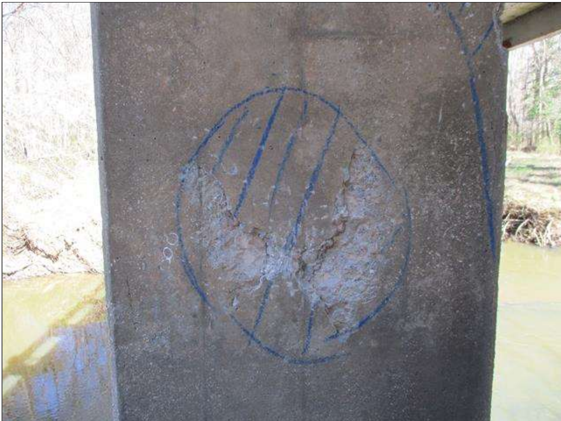
Bent 6 Pile 1: AT 5' DOWN FROM THE CAP, APPROXIMATELY 3 SQUARE FEET MAP CRACKING TO 1/16" WIDE WITH ASSOCIATED SPALLIN TO 1" DEEP AND DELAMINATION
