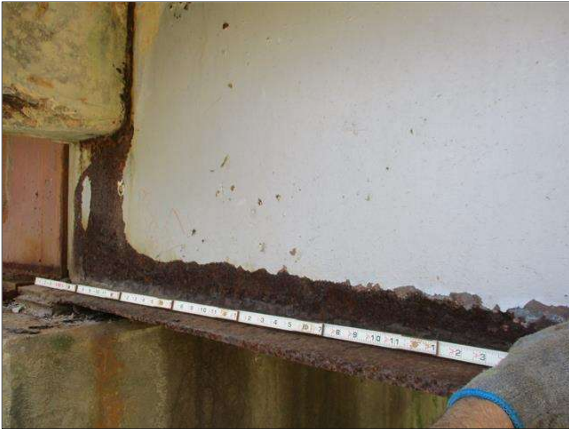
Span 8 Beam 4: [PROMPT ACTION REQUEST] BEAM END AT BENT 7, WEB, FULL HEIGHT, CORROSION WITH APPROXIMATELY 1/4" SECTION LOSS [AVERAGE 3/16" REMAINS] FOR 9" LONG, THEN IN THE LOWER 2" OF THE WEB, APPROXIMATELY 1/4" SECTION LOSS [AVERAGE 3/16" REMAINS] FOR 30" LONG
