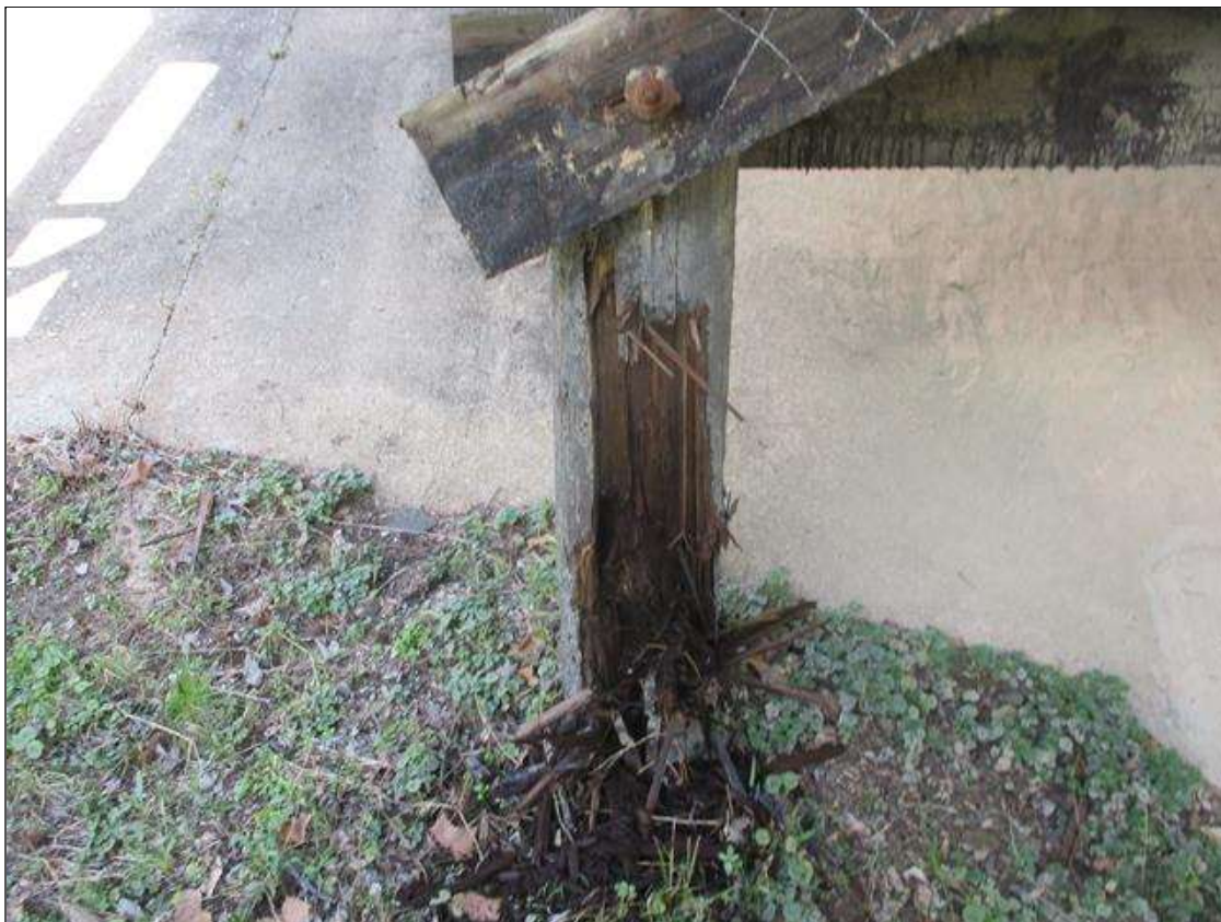
Bent 9 Pile 1: [PROMPT ACTION REQUEST] AT THE GROUNDLINE, DECAY AND SECTION LOSS WITH APPROXIMATELY 4" CORE REMAINING FOR APPROXIMATELY 4' HIGH
