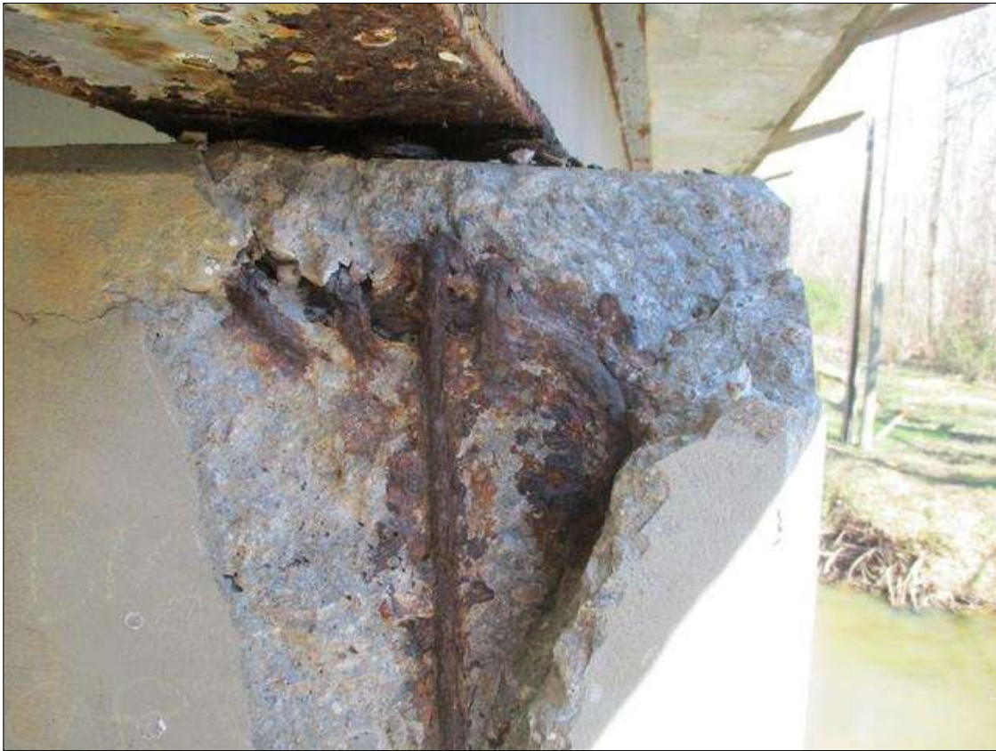
Bent 6 Cap 1: [PROMPT ACTION REQUEST] SOUTH FACE, RIGHT END, SPALLING WITH EXPOSED REBAR [APPROXIMATELY 2' LONG X FULL HEIGHT X UP TO 7" BACK X 3" DEEP]; SURFACE CORROSION AND PITTING TO 1/16" ON THE REBAR
