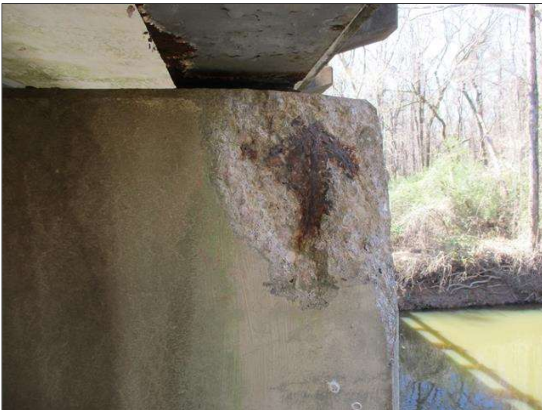
Bent 6 Cap 1: [PROMPT ACTION REQUEST] 19" X 14" X 5" DEEP SPALL WITH EXPOSED REBAR ON NORTH FACE UNDER GIRDER 1
