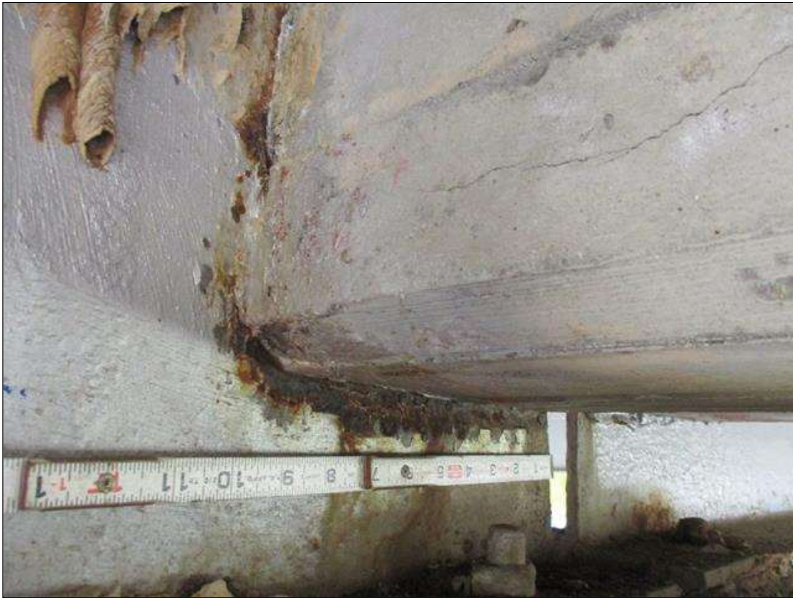
Span 3 Beam 2: [PROMPT ACTION REQUEST] BEAM END AT BENT 2, THERE IS AN APPROXIMATELY 1" WIDE BAND OF CORROSION THAT WRAPS THE REINFORCED CONCRETE DIAPHRAGM, APPROXIMATELY 1/4" SECTION LOSS [AVERAGE 1/16" REMAINS] FOR APPROXIMATELY 10" LONG.
