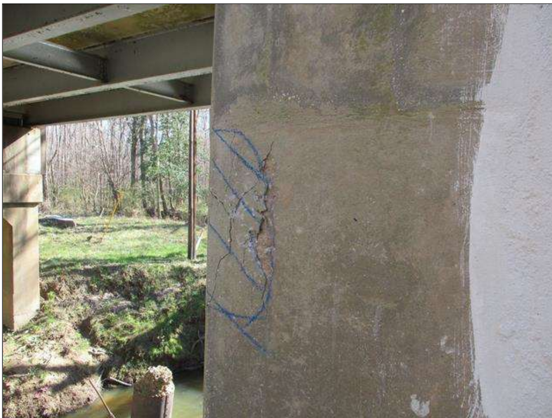
Bent 7 Pile 1: LEFT SIDE, APPROXIMATELY 2' DOWN FROM THE CAP, APPROXIMATELY 1 SQUARE FEET MAP CRACKING TO 1/8" WIDE WITH ASSOCIATED DELAMINATION AND SPALLING TO 3/4" DEEP
