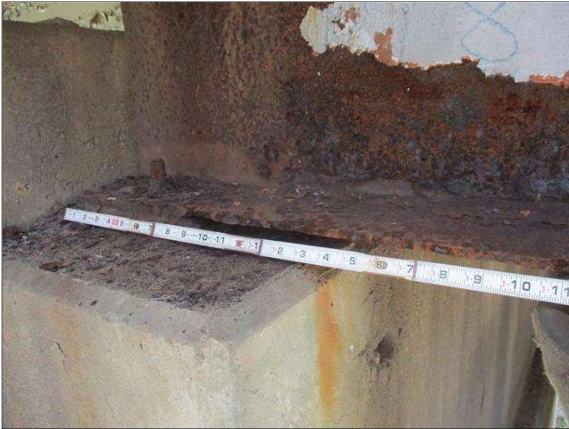
Span 8 Beam 1: [PROMPT ACTION REQUEST] BEAM END AT BENT 8, LOWER FLANGE, CORROSION WITH APPROXIMATELY 5/16" SECTION LOSS [AVERAGE 5/16" REMAINS] FOR APPROXIMATELY 2' LONG
