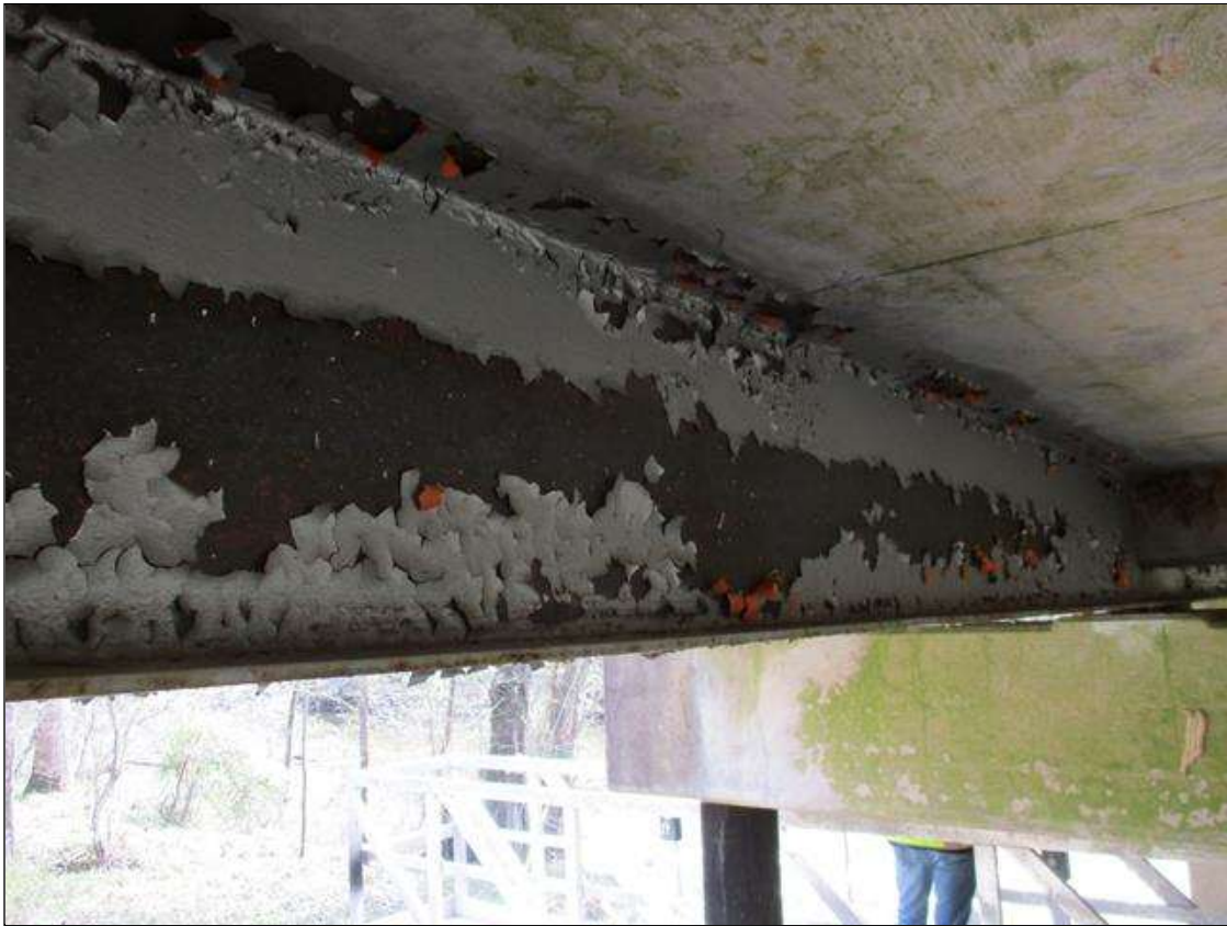
SUPERSTRUCTURE: VIEW OF TYPICAL PROTECTIVE COATING FAILURE
