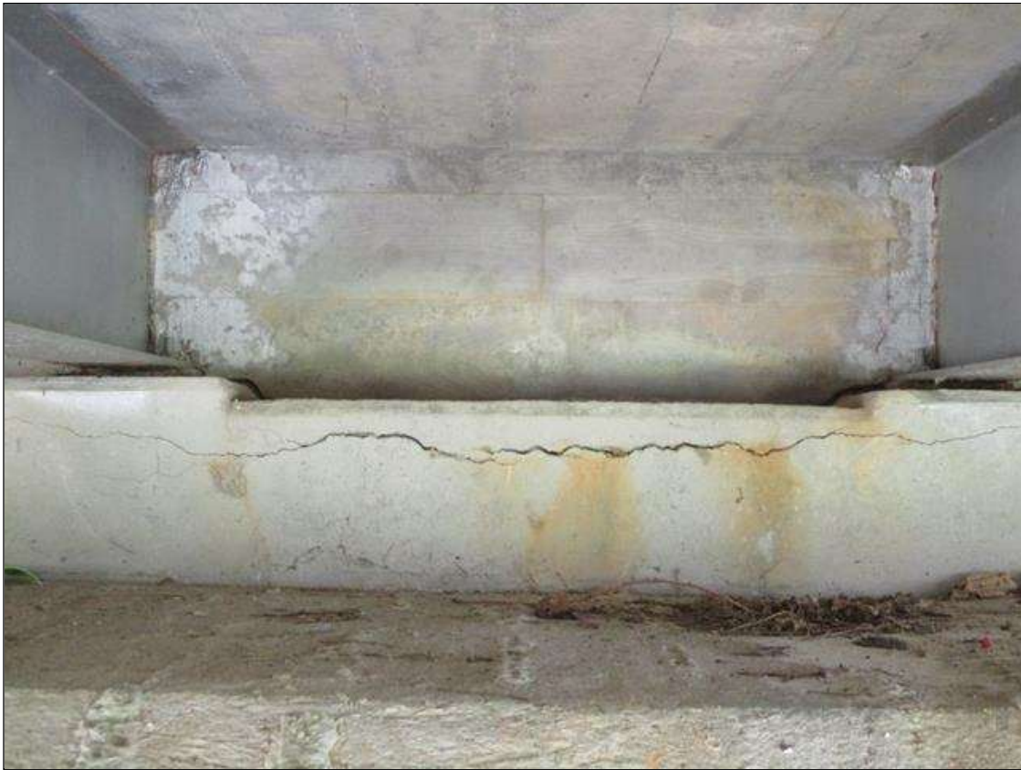
End Bent 1 Cap 1: CAP FACE AT BAY 2, UP TO 1/4" HORIZONTAL CRACKING
