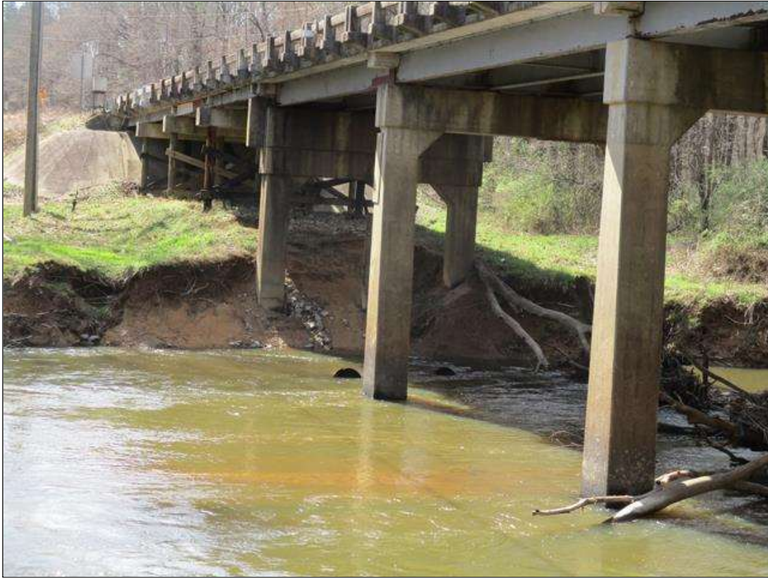
THE SOUTH AND NORTH BANKS HAVE EROSION WITH SLOUGHING [SOUTH APPROXIMATELY 100' LONG X UP TO 10' WIDE X UP TO 10' DEEP, AND NORTH APPROXIMATELY 50' LONG X UP TO 40' WIDE X UP TO 10' DEEP]
