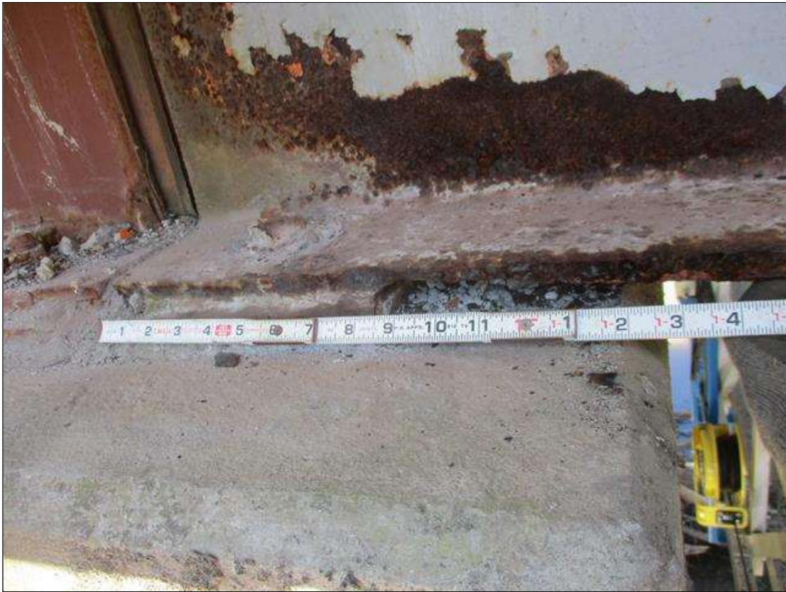
Span 6 Beam 4: [PROMPT ACTION REQUEST] BEAM END AT BENT 5, LOWER FLANGE, CORROSION WITH APPROXIMATELY 5/16" SECTION LOSS [AVERAGE 5/16" REMAINS] FOR APPROXIMATELY 12" LONG
