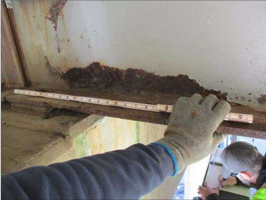
Span 6 Beam 3: [PROMPT ACTION REQUEST] 8" OUT FROM THE BEAM END AT BENT 5, IN THE LOWER 2" OF THE WEB, CORROSION WITH APPROXIMATELY 1/4" SECTION LOSS [AVERAGE 3/16" REMAINS] FOR 18" LONG.
