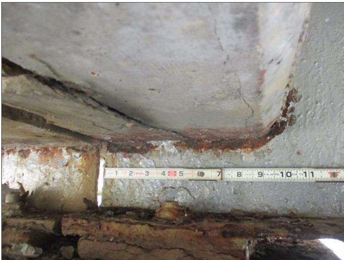
Span 1 Beam 4: [PROMPT ACTION REQUEST] BEAM END AT BENT 2, THERE IS AN APPROXIMATELY 1" WIDE BAND OF CORROSION THAT WRAPS THE REINFORCED CONCRETE DIAPHRAGM, 100% SECTION LOSS FOR APPROXIMATELY 2" LONG, THEN APPROXIMATELY 1/8" SECTION LOSS [AVERAGE 3/16" REMAINS] FOR APPROXIMATELY 8" LONG.
