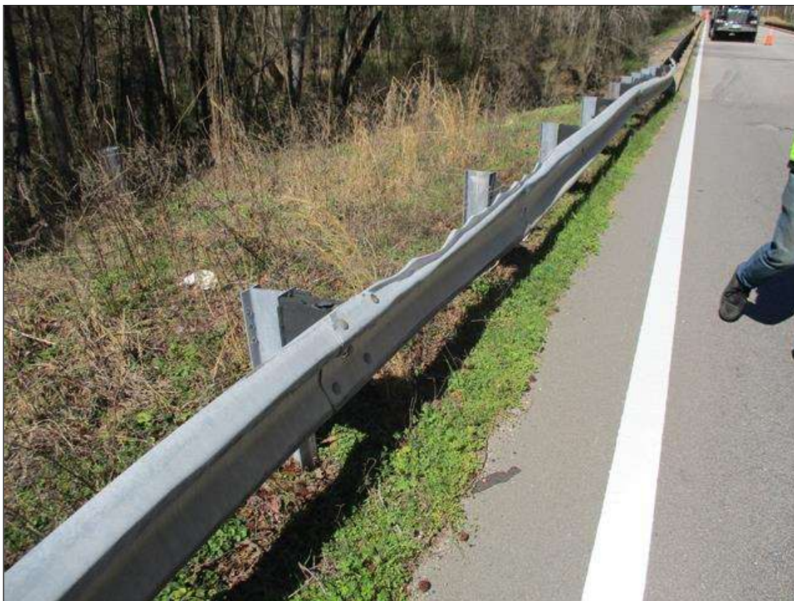
GUIDERAIL AT THE APPROACHES HAS BEEN "RUBBED" IN SCATTERED LOCATIONS, BUT IS GENERALLY SECURE AND FUNCTIONING.
