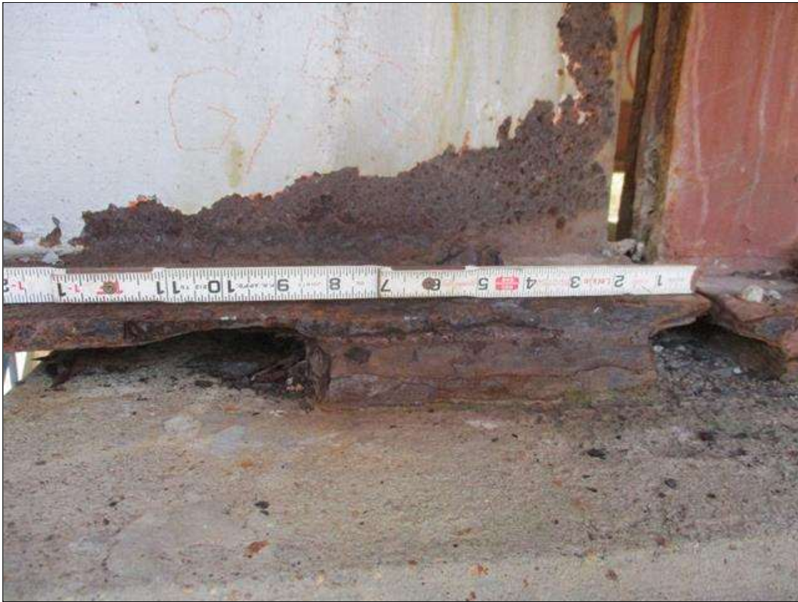
Span 6 Beam 1: [PROMPT ACTION REQUEST] BEAM END AT BENT 5, LOWER FLANGE, CORROSION WITH APPROXIMATELY 3/8" SECTION LOSS [AVERAGE 1/4" REMAINS] FOR APPROXIMATELY 12" LONG
