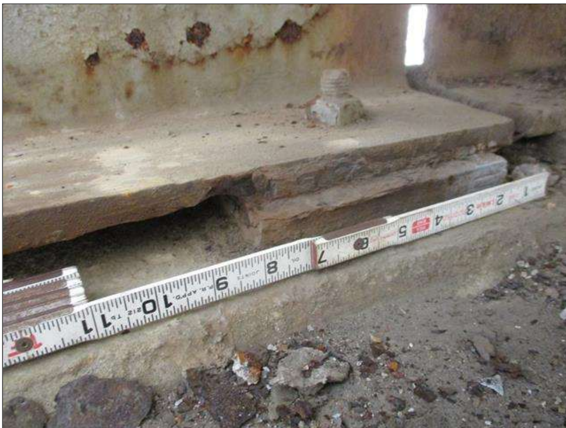
Span 5 Beam 3: [PROMPT ACTION REQUEST] 8" OUT FROM THE BEAM END AT BENT 5, LOWER FLANGE, CORROSION WITH APPROXIMATELY 1/4" SECTION LOSS [AVERAGE 3/8" REMAINS] FOR APPROXIMATELY 4" LONG
