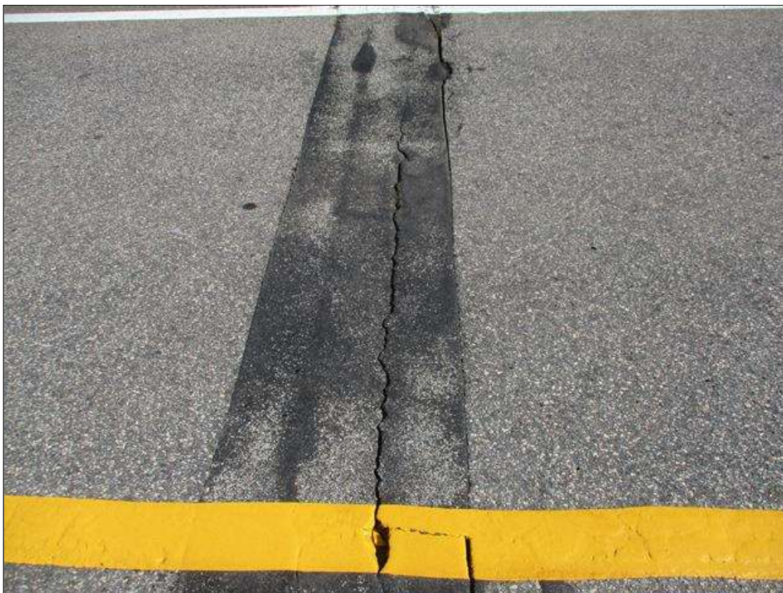
Expansion Joint : SCATTERED ALONG THE LENGTH, LONGITUDINAL CRACKING TO 2" WIDE
