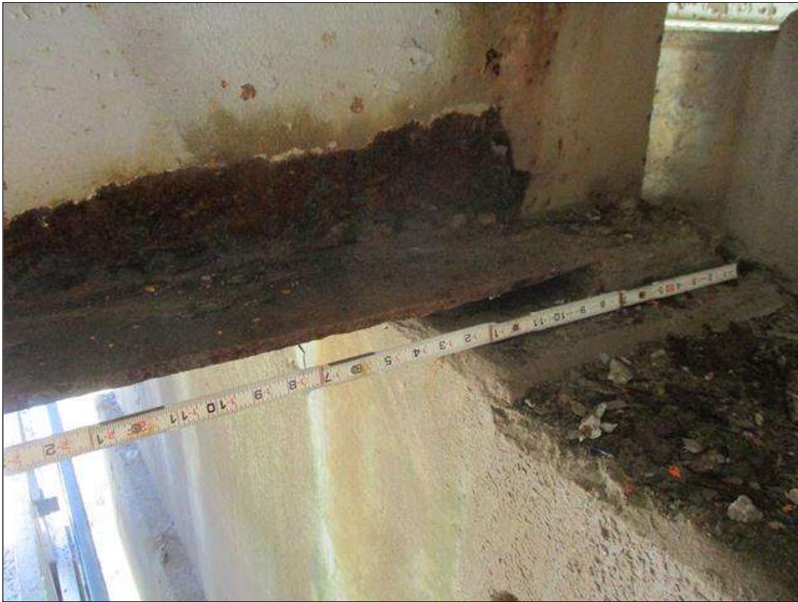
Span 8 Beam 2: [PROMPT ACTION REQUEST] BEAM END AT BENT 8, LOWER FLANGE, CORROSION WITH APPROXIMATELY 3/8" SECTION LOSS [AVERAGE 1/4" REMAINS] FOR APPROXIMATELY 1' LONG, THEN 1/4" SECTION LOSS [AVERAGE 3/8" REMAINS] FOR 2' LONG.
