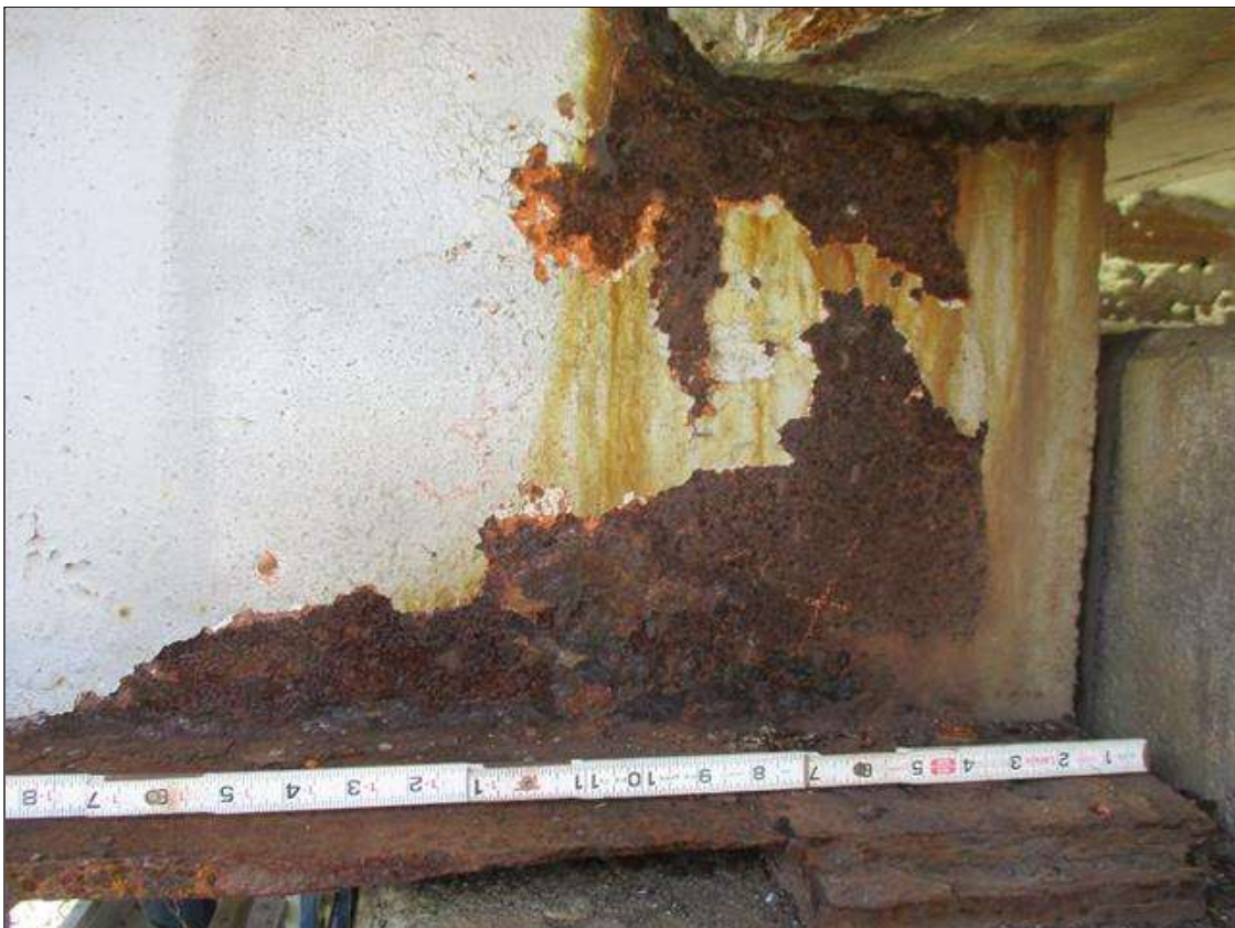
Span 8 Beam 4: [PROMPT ACTION REQUEST] BEAM END AT BENT 8, WEB, LOWER 3", CORROSION WITH APPROXIMATELY 1/8" SECTION LOSS [AVERAGE 5/16" REMAINS] FOR 18" LONG
