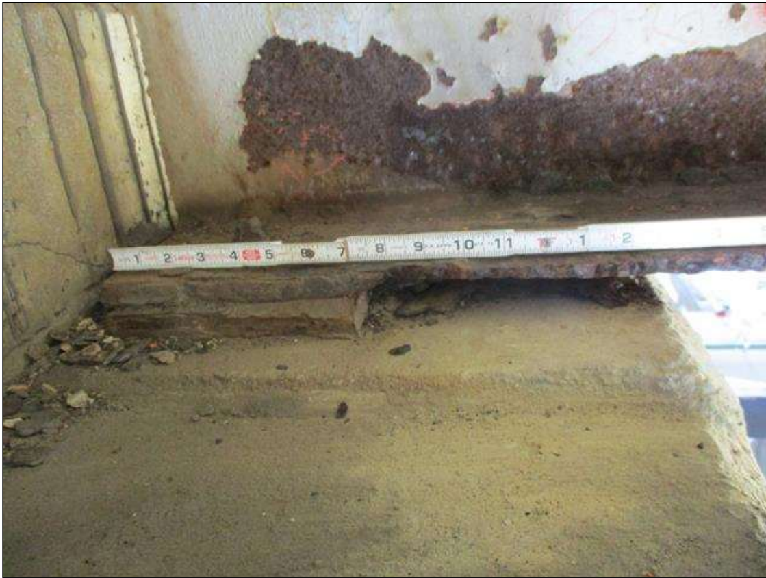
Span 5 Beam 3: [PROMPT ACTION REQUEST] BEAM END AT BENT 4, LOWER FLANGE, CORROSION WITH APPROXIMATELY 5/16" SECTION LOSS [AVERAGE 5/16" REMAINS] FOR APPROXIMATELY 15" LONG
