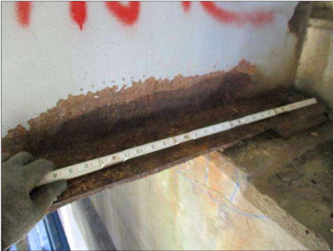
Span 5 Beam 2: [PROMPT ACTION REQUEST] 8" OUT FROM THE BEAM END AT BENT 4, IN THE LOWER 3" OF THE WEB, CORROSION WITH APPROXIMATELY 3/16" SECTION LOSS [AVERAGE 1/4" REMAINS] FOR 18" LONG.
