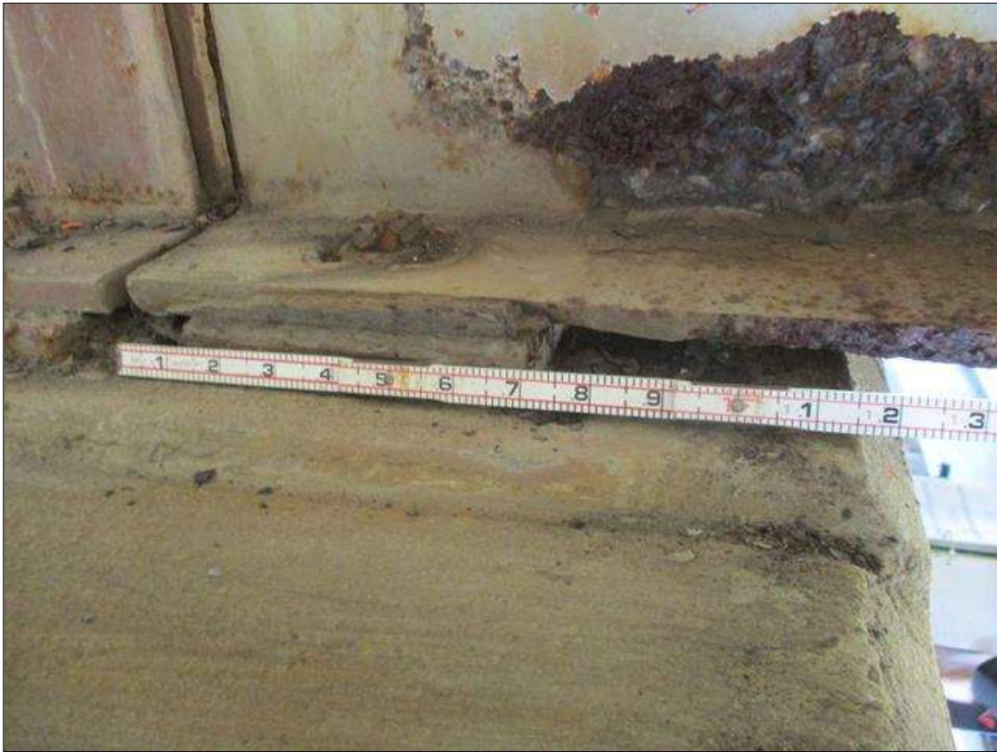
Span 6 Beam 3: [PROMPT ACTION REQUEST] BEAM END AT BENT 5, LOWER FLANGE, CORROSION WITH APPROXIMATELY 3/16" SECTION LOSS [AVERAGE 7/16" REMAINS] FOR APPROXIMATELY 12" LONG
