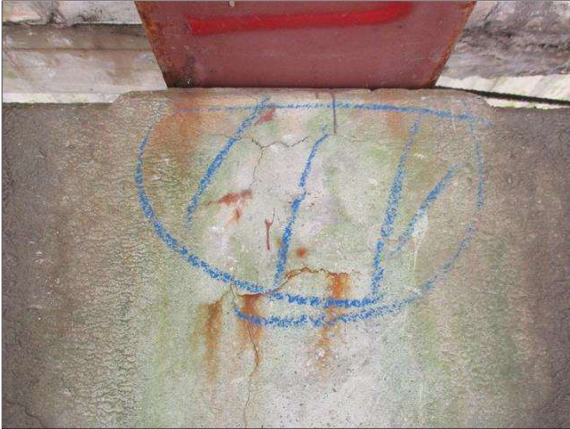
Bent 5 Cap 1: SOUTH FACE AT BEAM 2, TOP, APPROXIMATELY 1 SQUARE FEET MAP CRACKING TO 1/16" WIDE WITH ASSOCIATED DELAMINATION
