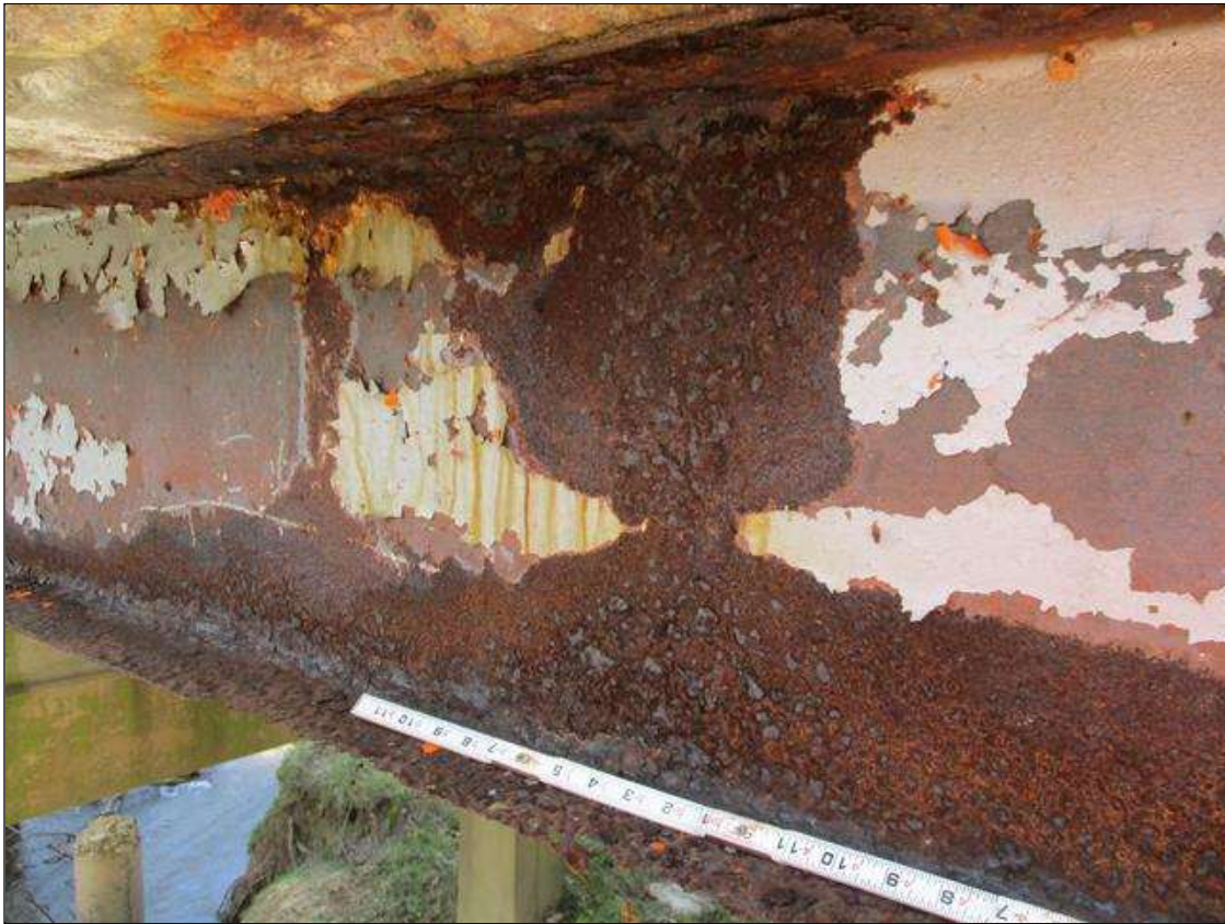
Span 9 Beam 6: [PROMPT ACTION REQUEST] APPROXIMATELY 5.5' OUT FROM THE BEAM END AT BENT 9, WEB, FULL HEIGHT, CORROSION WITH APPROXIMATELY 5/16" SECTION LOSS [AVERAGE 1/8" REMAINS] FOR 3" LONG. APPROXIMATELY 2' OUT FROM THE BEAM END AT BENT 9, WEB, LOWER AND UPPER 1", CORROSION WITH APPROXIMATELY 5/16" SECTION LOSS [AVERAGE 1/8" REMAINS] FOR 12" LONG.
