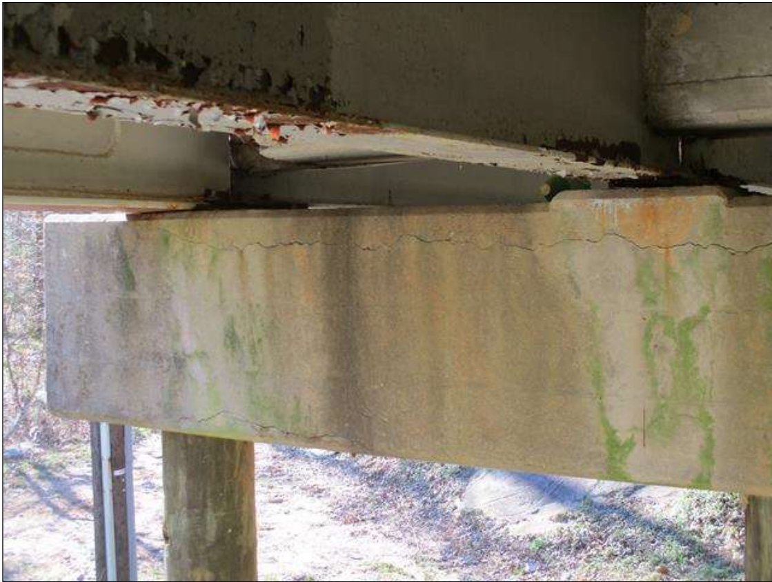
Bent 2 Cap 1: NORTH FACE, APPROXIMATELY 4" DOWN FROM THE TOP BETWEEN BEAMS 2-6, HORIZONTAL CRACKING TO 3/16" WIDE WITH ASSOCIATED DELAMINATION ABOVE, AND LOWER 6" OF THE NORTH FACE, SCATTERED HORIZONTAL CRACKING TO 1/16" WIDE
