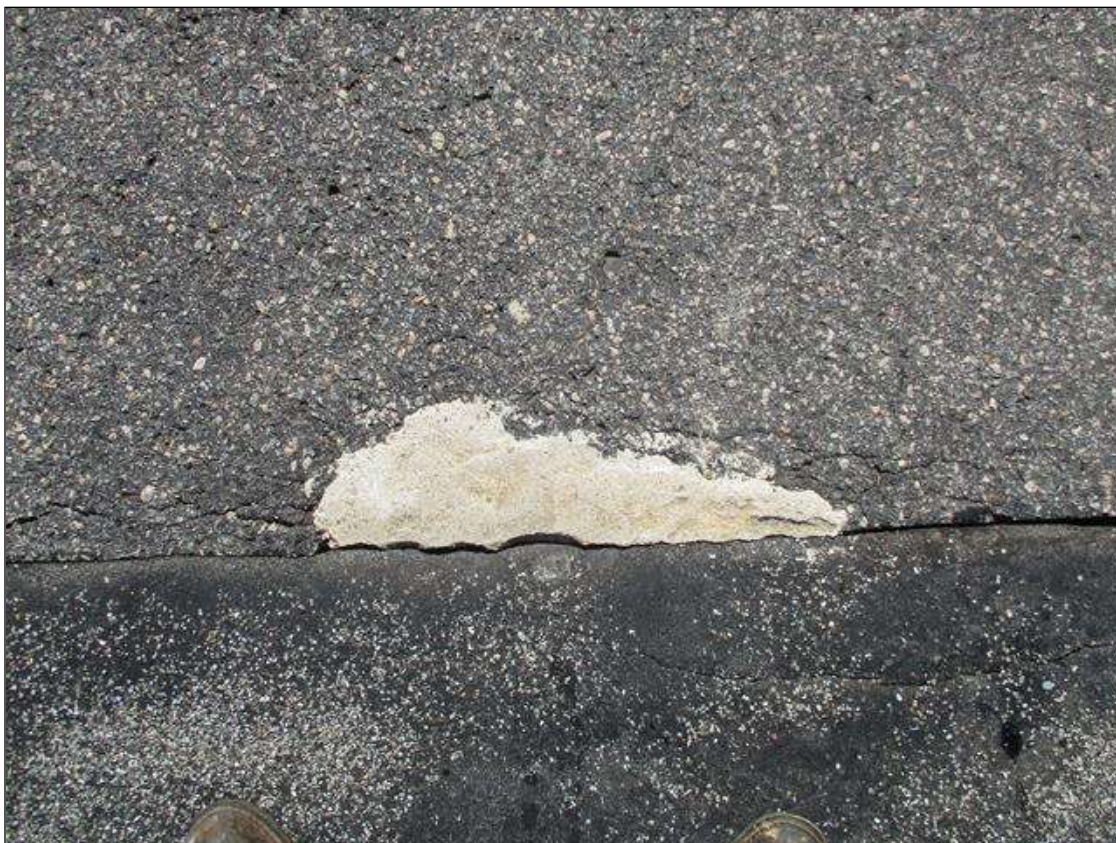
Span 5 Wearing Surface: RIGHT LANE AT BENT 5, APPROXIMATELY 1 SQUARE FEET SOUND PATCHING
