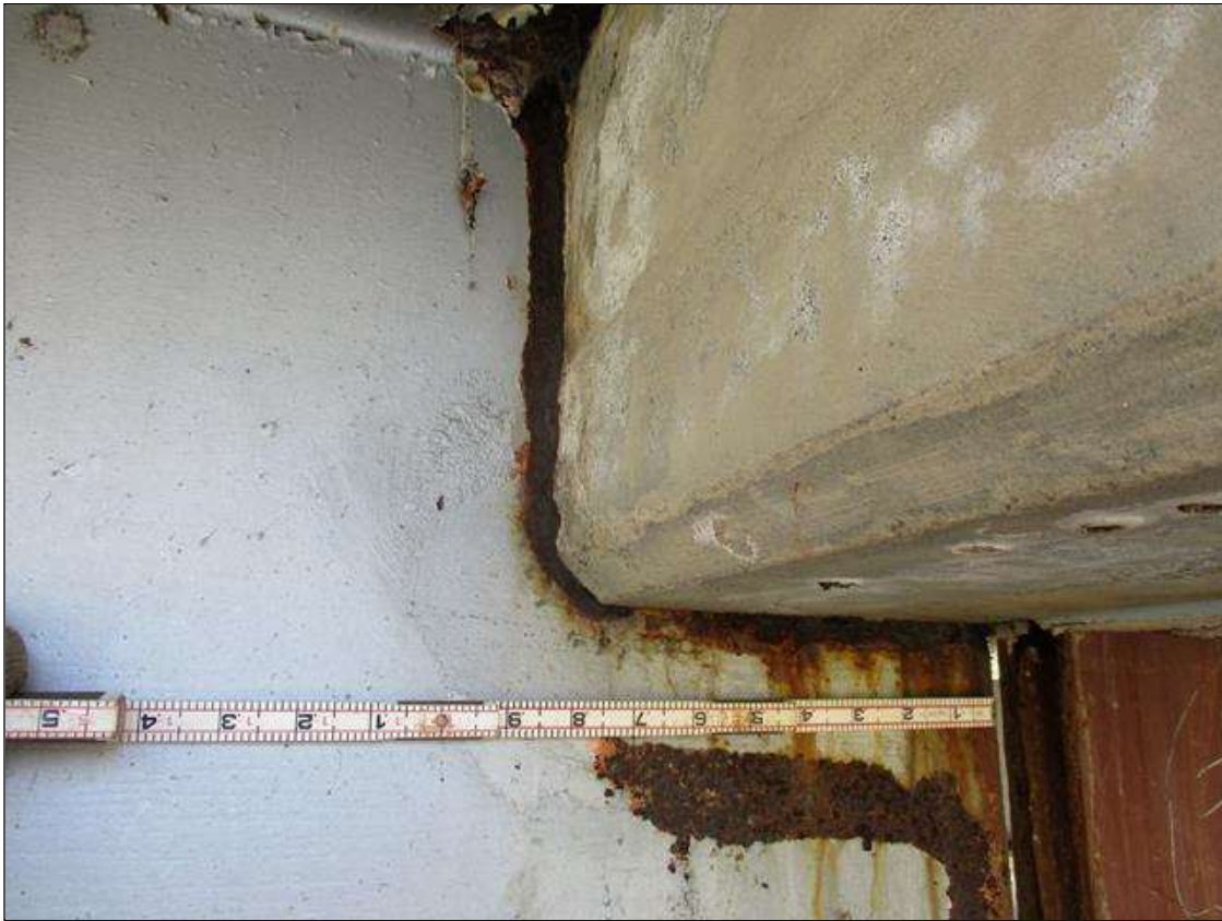
Span 6 Beam 1: [PROMPT ACTION REQUEST] BEAM END AT BENT 5, THERE IS AN APPROXIMATELY 1" WIDE BAND OF CORROSION THAT WRAPS THE REINFORCED CONCRETE DIAPHRAGM, APPROXIMATELY 3/16" SECTION LOSS [AVERAGE 1/4" REMAINS] FOR APPROXIMATELY 10" LONG.
