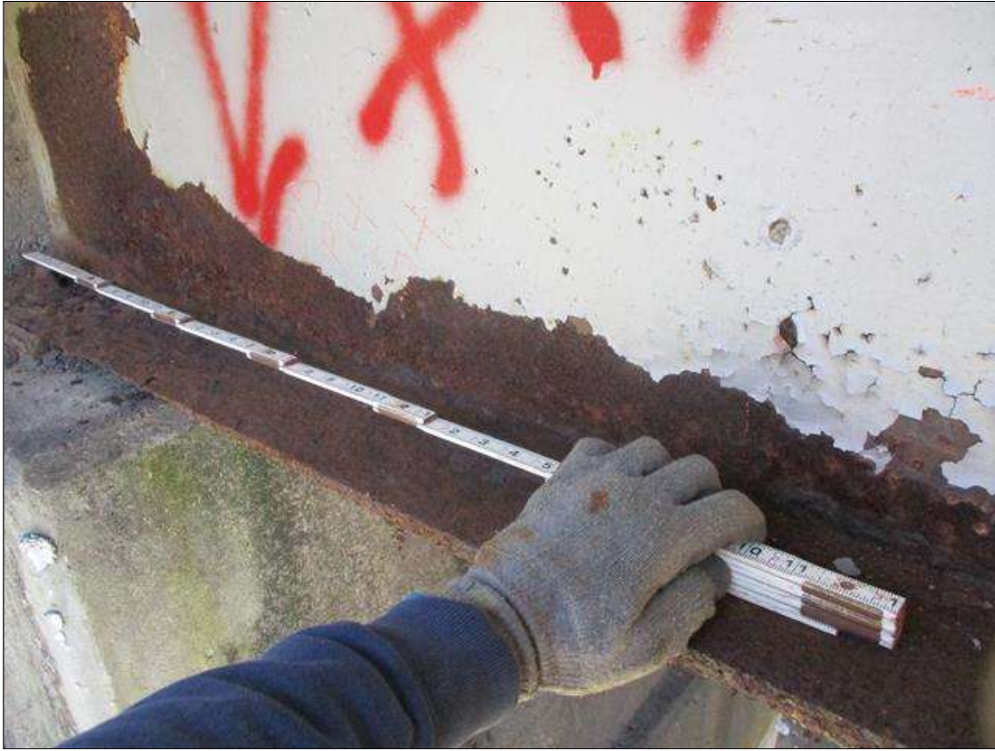
Span 5 Beam 4: [PROMPT ACTION REQUEST] 8" OUT FROM THE BEAM END AT BENT 4, IN THE LOWER 3" OF THE WEB, CORROSION WITH APPROXIMATELY 5/16" SECTION LOSS [AVERAGE 1/8" REMAINS] FOR 30" LONG.
