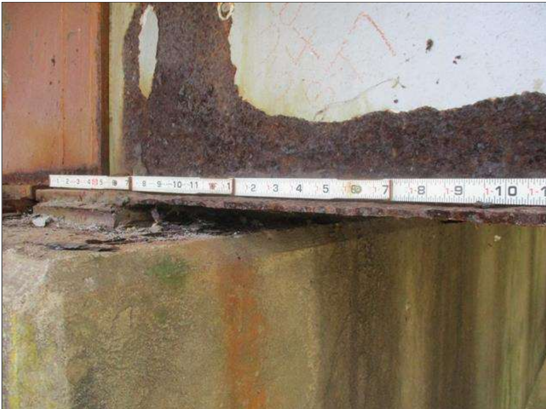
Span 8 Beam 4: [PROMPT ACTION REQUEST] BEAM END AT BENT 7, LOWER FLANGE, CORROSION WITH APPROXIMATELY 3/8" SECTION LOSS [AVERAGE 1/4" REMAINS] FOR APPROXIMATELY 2' LONG.
