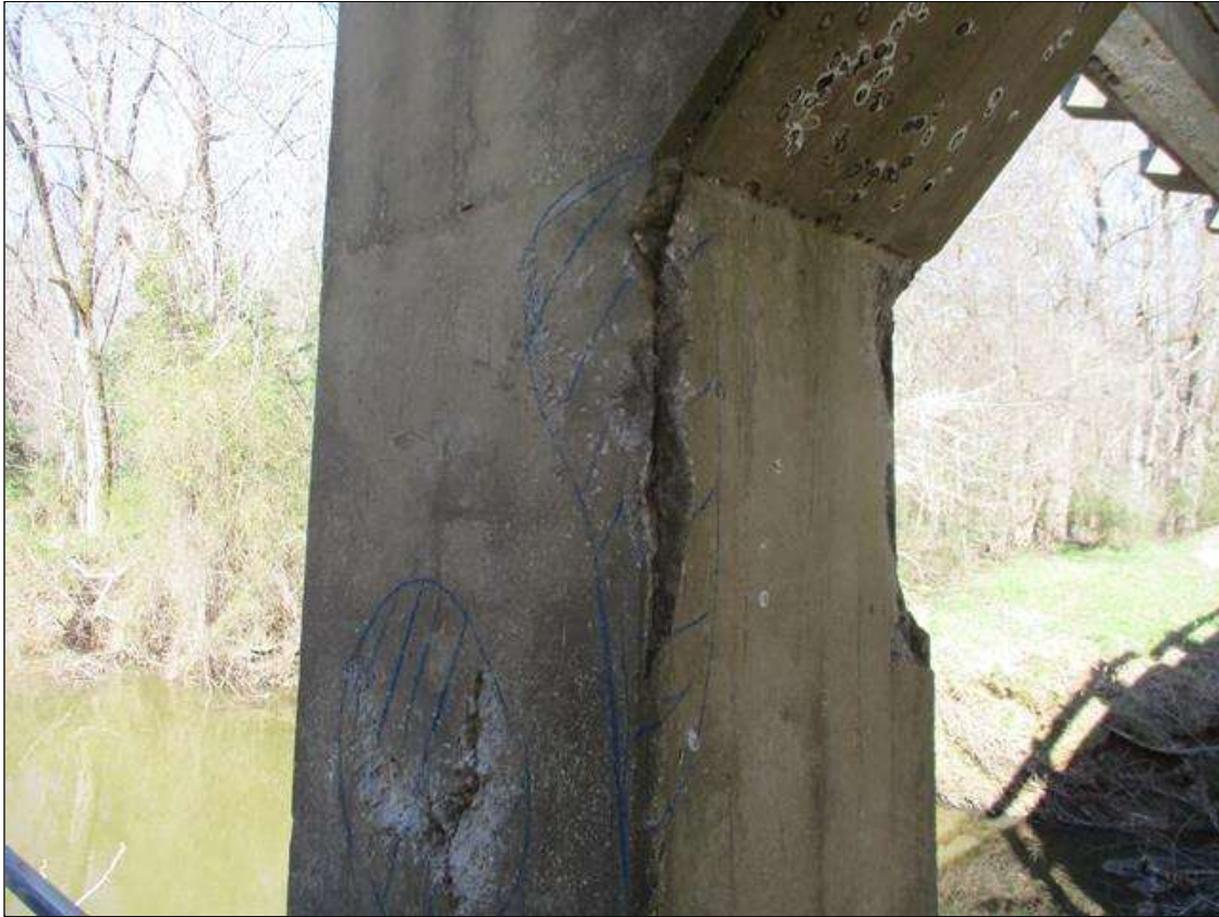
Bent 6 Pile 1: AT 4' DOWN FROM THE CAP, APPROXIMATELY 3 SQUARE FEET MAP CRACKING TO 1/16" WIDE WITH ASSOCIATED SPALLIN TO 2" DEEP AND DELAMINATION
