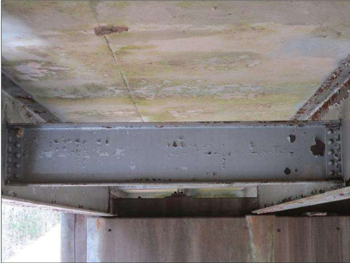
STEEL DIAPHRAGMS: FRECKLED CORROSION AND SCATTERED CORROSION IN AREAS OF PROTECTIVE COATING FAILURE
