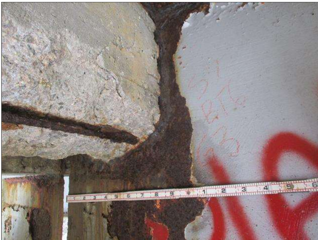
Span 7 Beam 3: [PROMPT ACTION REQUEST] BEAM END AT BENT 6, THERE IS AN APPROXIMATELY 2" WIDE BAND OF CORROSION THAT WRAPS THE REINFORCED CONCRETE DIAPHRAGM, APPROXIMATELY 1/4" SECTION LOSS [AVERAGE 3/16" REMAINS] FOR APPROXIMATELY 10" LONG.
