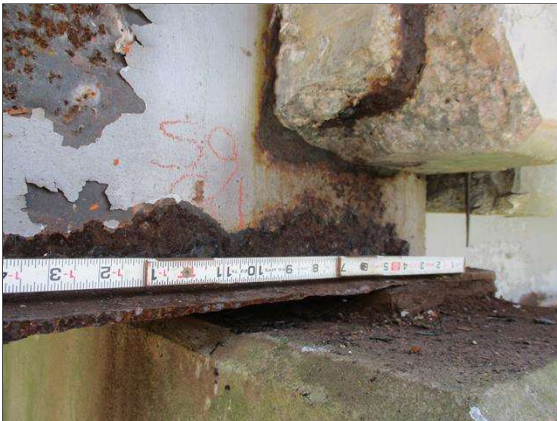
Span 9 Beam 1: [PROMPT ACTION REQUEST] BEAM END AT BENT 8, LOWER LEFT FLANGE, CORROSION WITH APPROXIMATELY 5/16" SECTION LOSS [AVERAGE 1/8" REMAINS] FOR APPROXIMATELY 15" LONG.
