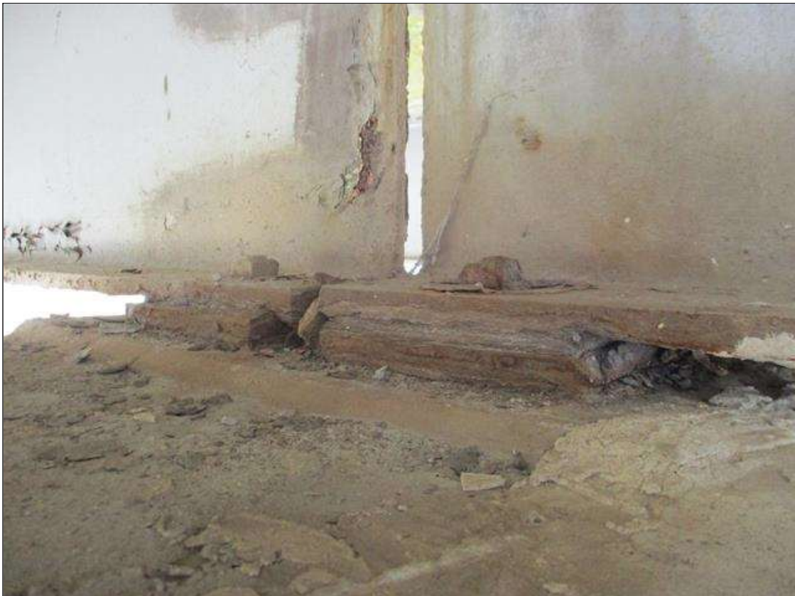
TYPICAL BEARING SURFACE CORROSION
