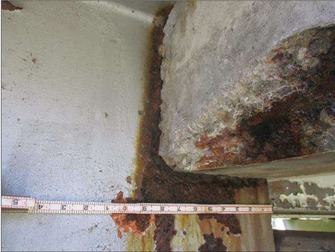
Span 8 Beam 4: [PROMPT ACTION REQUEST] BEAM END AT BENT 8, THERE IS AN APPROXIMATELY 1" WIDE BAND OF CORROSION THAT WRAPS THE REINFORCED CONCRETE DIAPHRAGM, APPROXIMATELY 1/4" SECTION LOSS [AVERAGE 3/16" REMAINS] FOR APPROXIMATELY 10" LONG.
