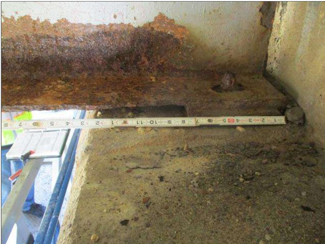
Span 5 Beam 2: [PROMPT ACTION REQUEST] BEAM END AT BENT 4, LOWER FLANGE, CORROSION WITH APPROXIMATELY 5/16" SECTION LOSS [AVERAGE 5/16" REMAINS] FOR APPROXIMATELY 18" LONG
