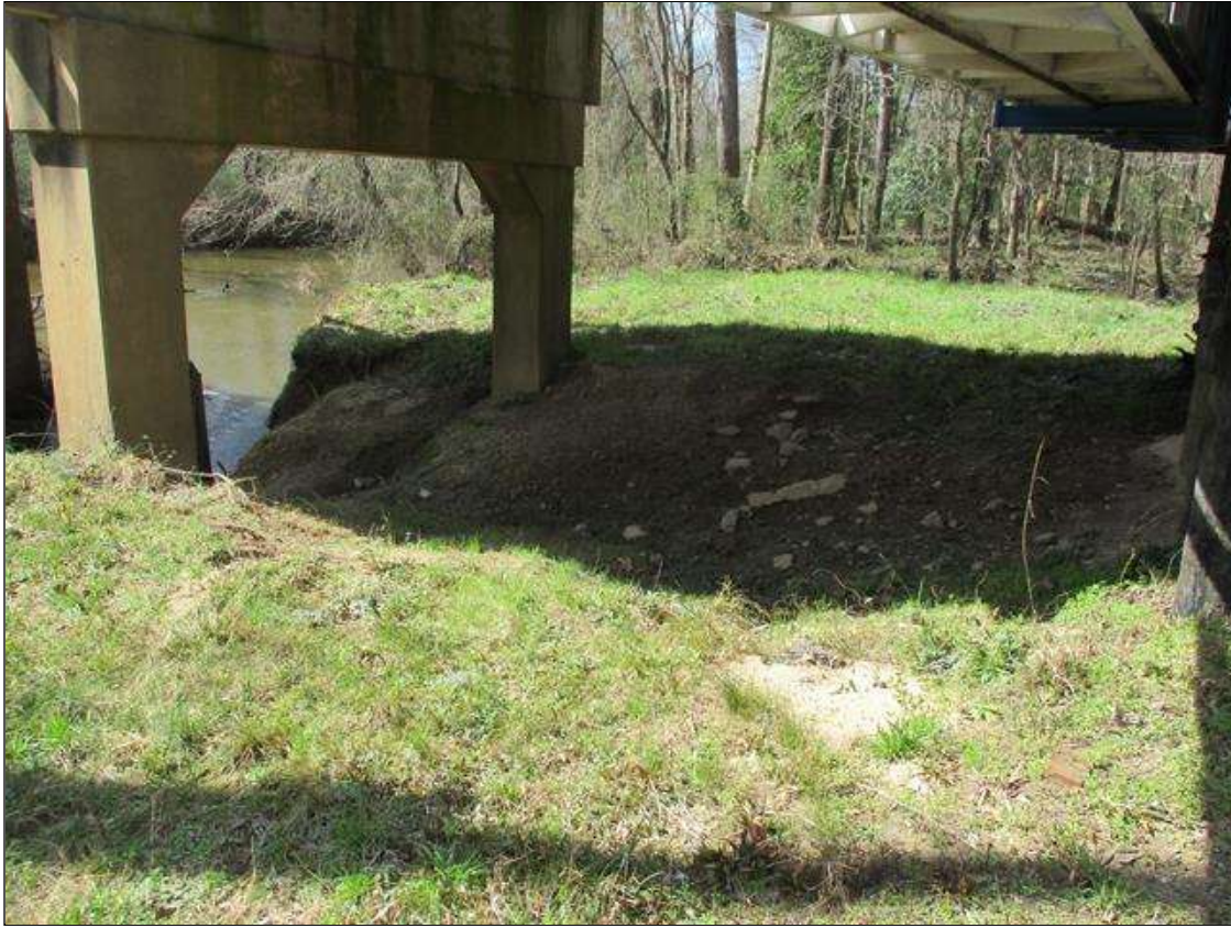
THE SOUTH AND NORTH BANKS HAVE EROSION WITH SLOUGHING [SOUTH APPROXIMATELY 100' LONG X UP TO 10' WIDE X UP TO 10' DEEP, AND NORTH APPROXIMATELY 50' LONG X UP TO 40' WIDE X UP TO 10' DEEP]
