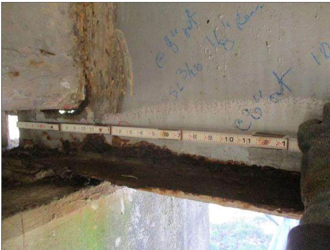
Span 3 Beam 1: [PROMPT ACTION REQUEST] APPROXIMATELY 8" OUT FROM THE BEAM END AT BENT 2, IN THE LOWER 1" OF THE WEB, CORROSION WITH APPROXIMATELY 3/16" SECTION LOSS [AVERAGE 1/8" REMAINS] FOR APPROXIMATELY 18" LONG.
