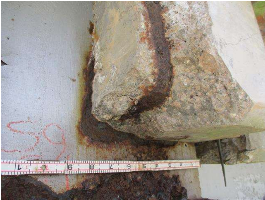
Span 9 Beam 1: [PROMPT ACTION REQUEST] BEAM END AT BENT 8, THERE IS AN APPROXIMATELY 1" WIDE BAND OF CORROSION THAT WRAPS THE REINFORCED CONCRETE DIAPHRAGM, APPROXIMATELY 3/16" SECTION LOSS [AVERAGE 3/16" REMAINS] FOR APPROXIMATELY 10" LONG.
