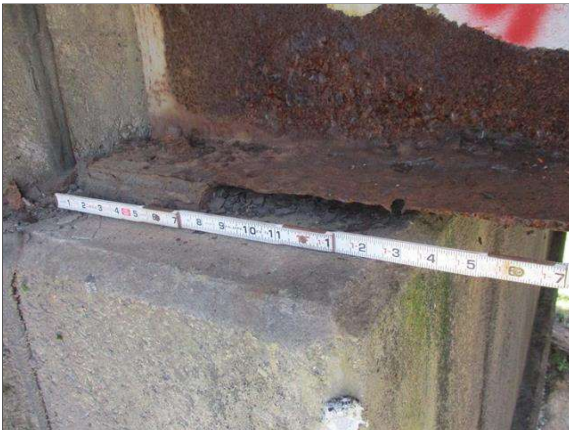
Span 5 Beam 4: [PROMPT ACTION REQUEST] BEAM END AT BENT 4, LOWER FLANGE, CORROSION WITH APPROXIMATELY 1/2" SECTION LOSS [AVERAGE 1/8" REMAINS] WITH KNIFE EDGING FOR APPROXIMATELY 15" LONG, THEN TAPERING TO FULL SECTION OVER THE NEXT 2' LONG
