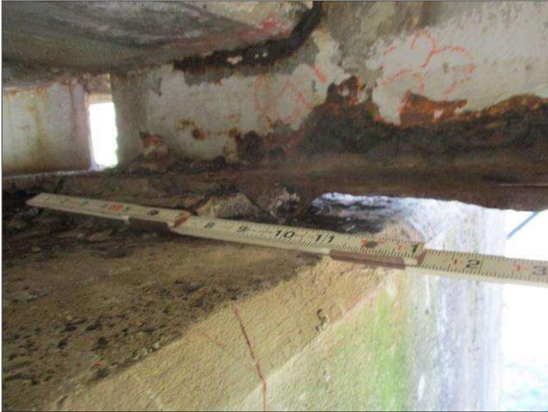
Span 3 Beam 1: [PROMPT ACTION REQUEST] APPROXIMATELY 6" OUT FROM THE BEAM END AT BENT 2, LOWER FLANGE, CORROSION WITH 100% SECTION LOSS FOR APPROXIMATELY 5" LONG, THEN TAPERING TO FULL SECTION OVER THE NEXT 5" [AVERAGE 3/16" REMAINS]
