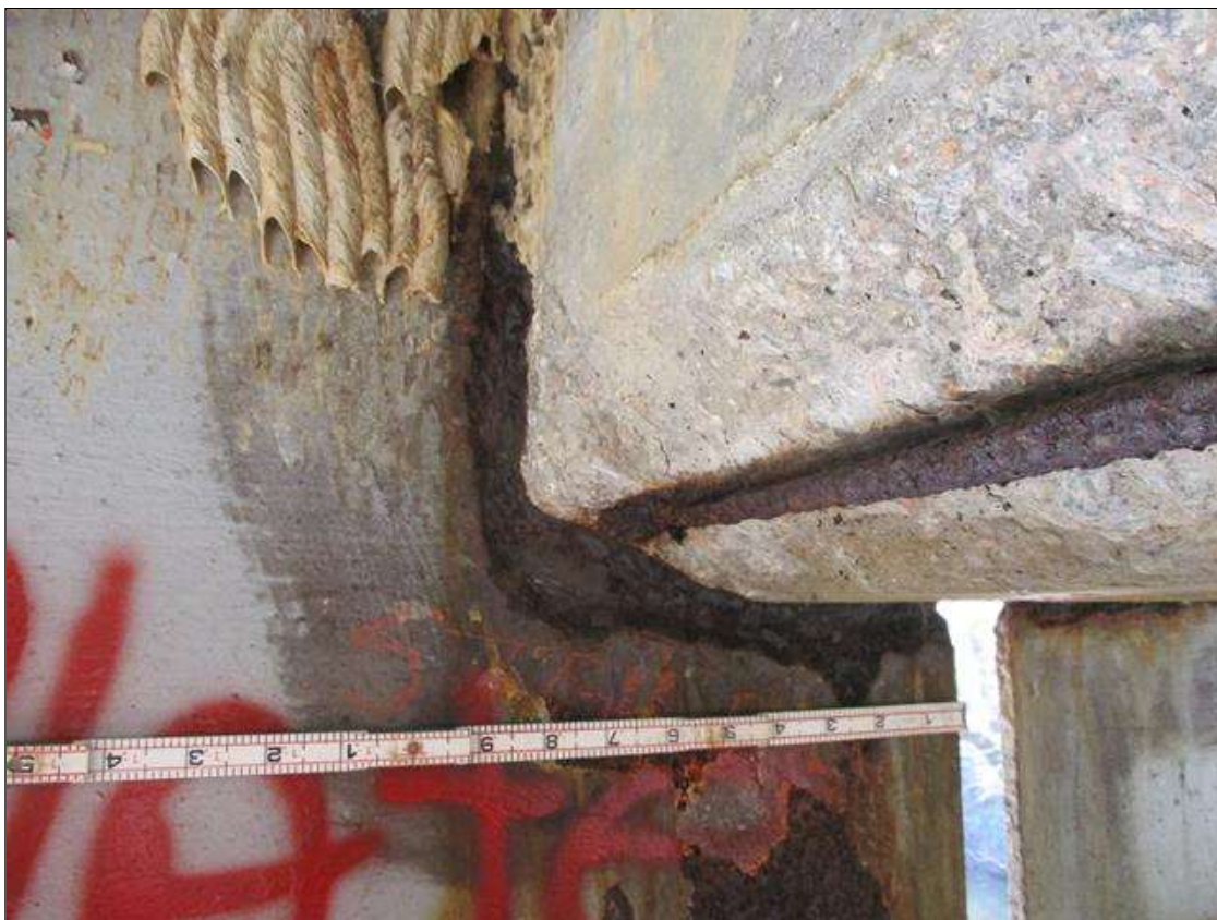
Span 7 Beam 4: [PROMPT ACTION REQUEST] BEAM END AT BENT 6, THERE IS AN APPROXIMATELY 2" WIDE BAND OF CORROSION THAT WRAPS THE REINFORCED CONCRETE DIAPHRAGM, APPROXIMATELY 3/8" SECTION LOSS [AVERAGE 1/16" REMAINS] FOR APPROXIMATELY 10" LONG.
