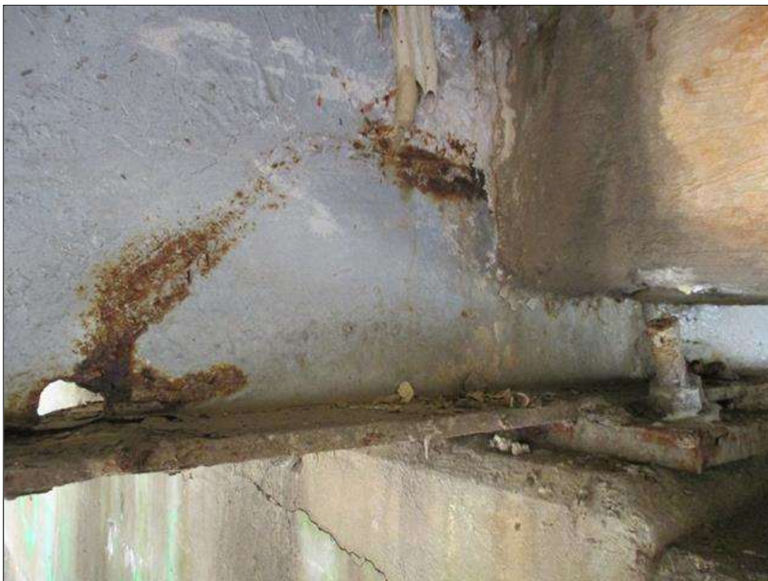
Span 3 Beam 3: [NEW REPAIR] BEAM END AT BENT 2 HAS BEEN SECTIONED, APPROXIMATELY 2' LONG X 7.5" WIDE X UP TO 8" HIGH
