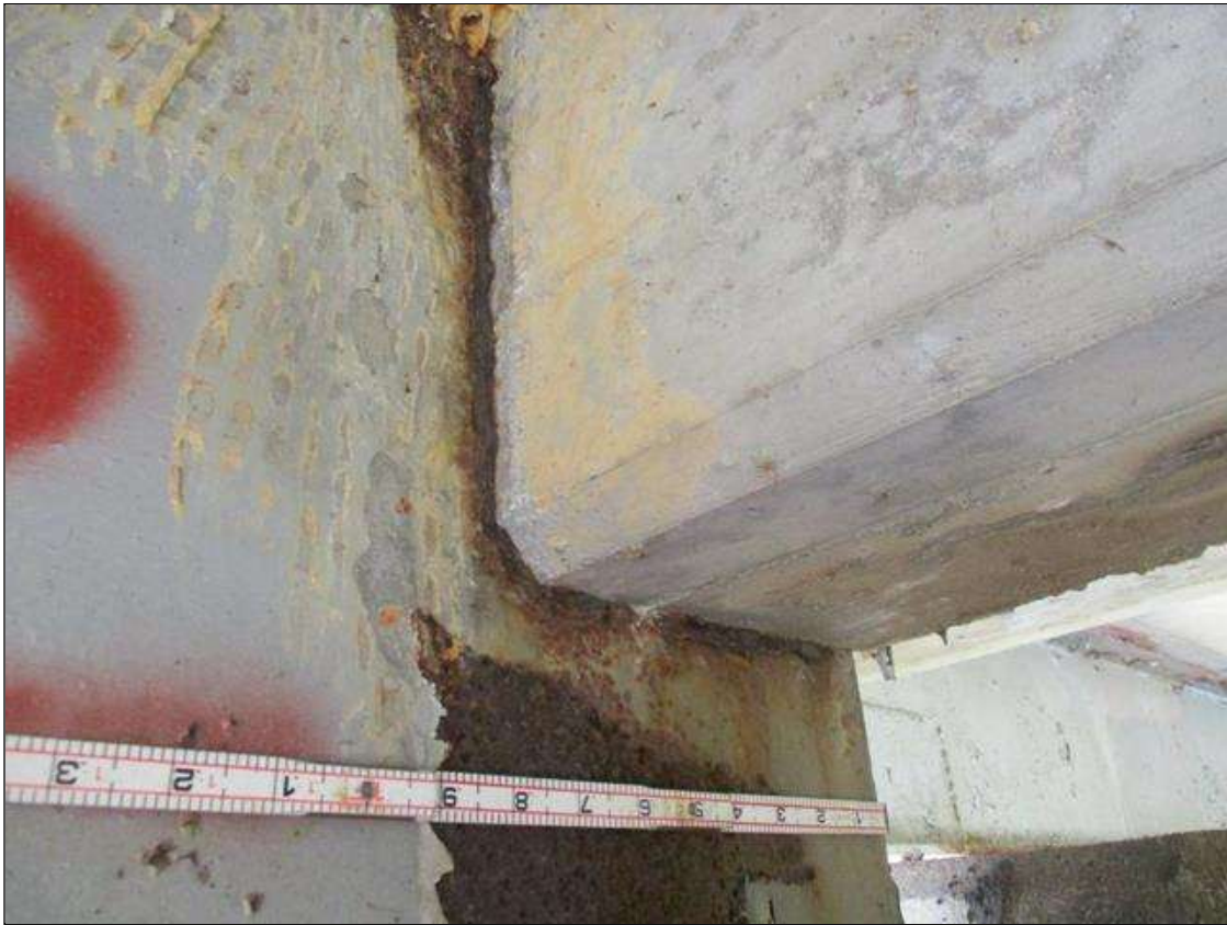
Span 5 Beam 4: [PROMPT ACTION REQUEST] BEAM END AT BENT 4, THERE IS AN APPROXIMATELY 1" WIDE BAND OF CORROSION THAT WRAPS THE REINFORCED CONCRETE DIAPHRAGM, APPROXIMATELY 1/8" SECTION LOSS [AVERAGE 5/16" REMAINS] FOR APPROXIMATELY 10" LONG.
