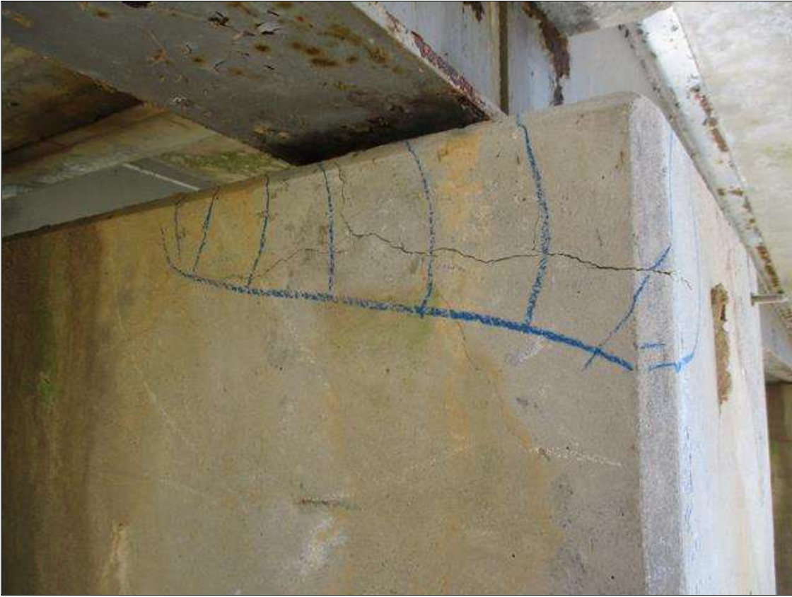
Bent 7 Cap 1: NORTH FACE, LEFT END, TOP CORNER, APPROXIMATELY 2 SQUARE FEET MAP CRACKING TO 1/32" WIDE WITH ASSOCIATED DELAMINATION
