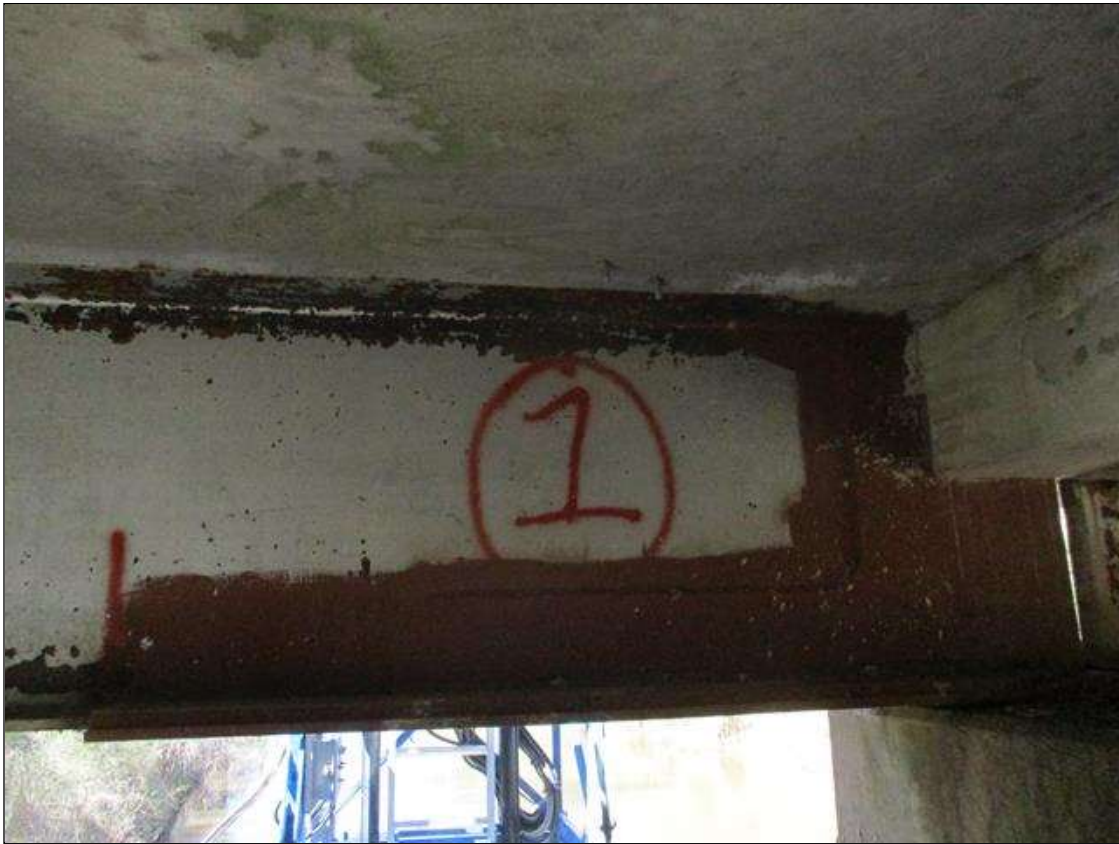
Span 5 Beam 1: [NEW REPAIR] BEAM END AT BENT 5, PLATES HAVE BEEN WELDED TO BOTH SIDES OF THE WEB [4' LONG X UP TO FULL HEIGHT] AND ON THE UPPER AND LOWER SIDES OF THE LOWER FLANGE [5.33' LONG X 1' WIDE] IN THE AREAS OF PAST SECTION LOSS.
