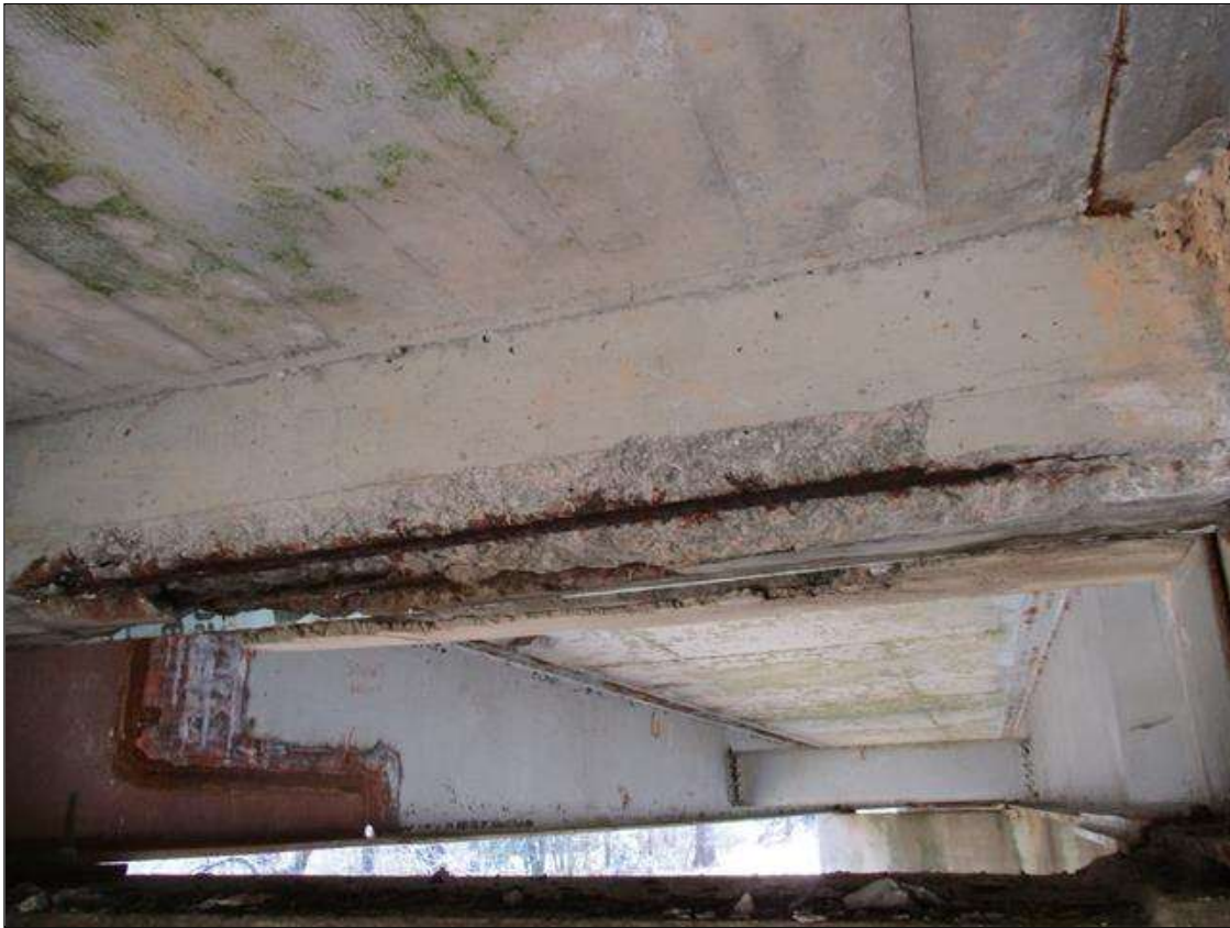
Span 8 Beam 2: [PROMPT ACTION REQUEST] BAY 3 AT BENT 7, REINFORCED CONCRETE DIAPHRAGM, SPALLING WITH EXPOSED REBAR [APPROXIMATELY 5' LONG X 10" WIDE X UP TO 3" DEEP]. THE REBAR IS DELAMINATED FROM THE CONCRETE AND HAS SURFACE CORROSION AND PITTING UP TO 1/16" DEEP.
