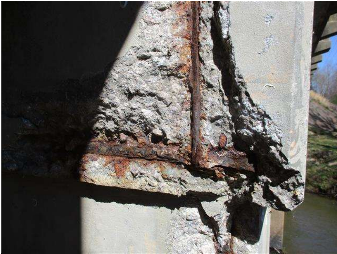
Bent 6 Cap 1: [PROMPT ACTION REQUEST] SOUTH FACE, RIGHT END, SPALLING WITH EXPOSED REBAR [APPROXIMATELY 2' LONG X FULL HEIGHT X UP TO 7" BACK X 3" DEEP]; SURFACE CORROSION AND PITTING TO 1/16" ON THE REBAR
