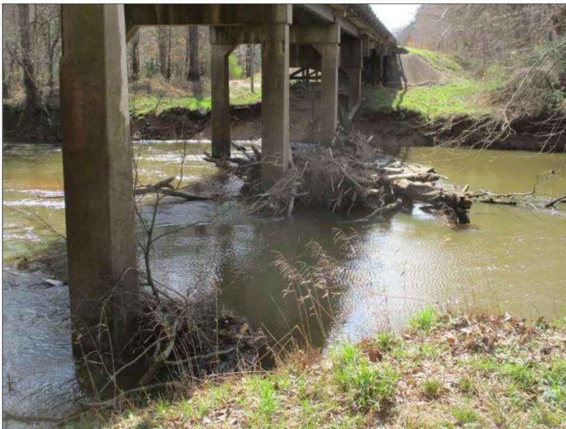
UPSTREAM OF BENTS 4-7, DRIFT COLLECTED [APPROXIMATELY 120 CUBIC YARDS TOTAL]
