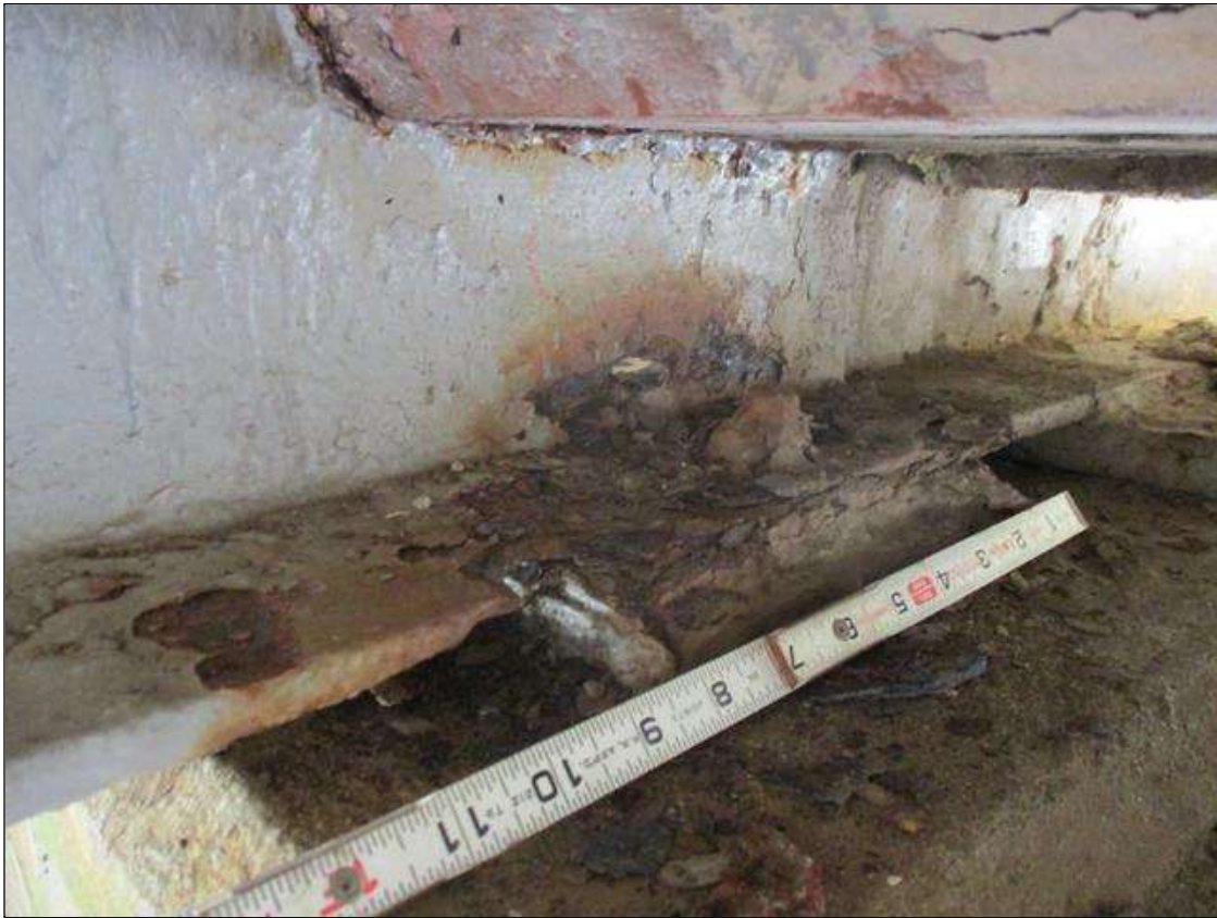
Span 1 Beam 3: [PROMPT ACTION REQUEST] BEAM END AT BENT 2, LOWER LEFT FLANGE, CORROSION WITH APPROXIMATELY 1/4" SECTION LOSS [AVERAGE 1/8" REMAINS] FOR APPROXIMATELY 11" LONG, AND LOWER RIGHT FLANGE, CORROSION WITH 100% SECTION LOSS FOR APPROXIMATELY 11" LONG
