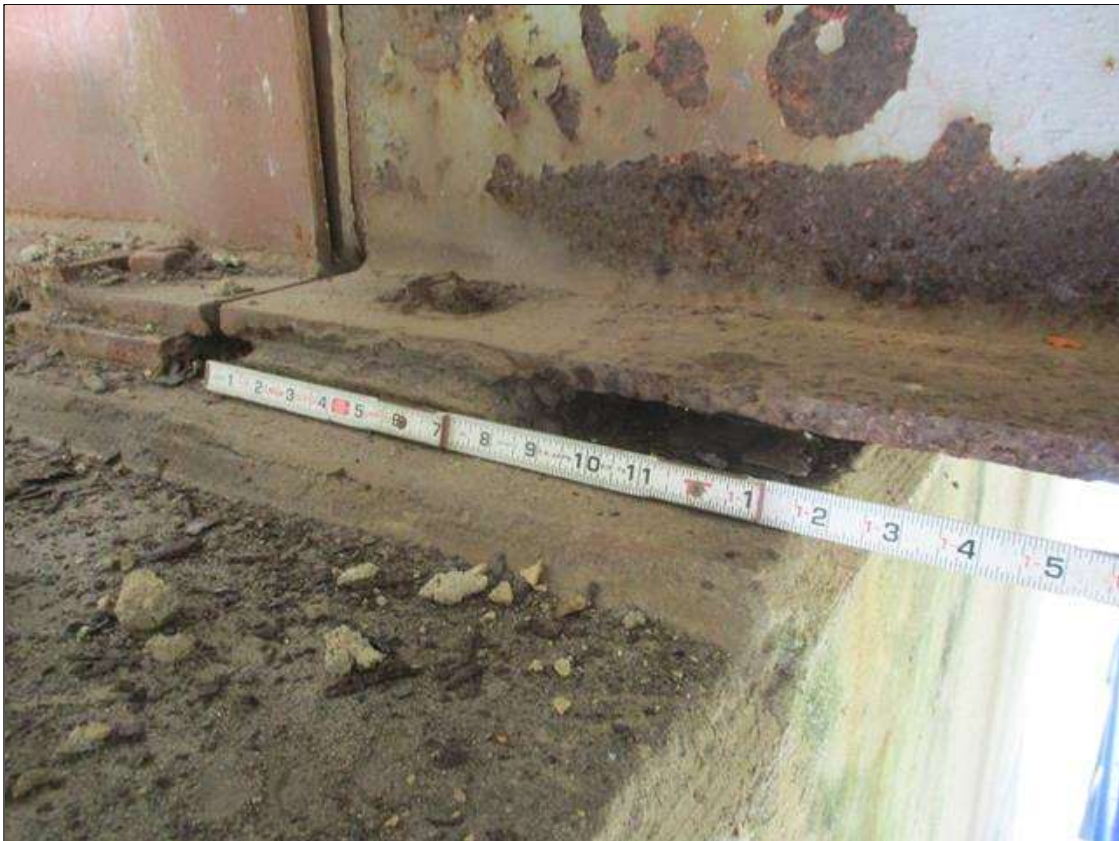
Span 6 Beam 2: [PROMPT ACTION REQUEST] BEAM END AT BENT 5, LOWER FLANGE, CORROSION WITH APPROXIMATELY 1/8" SECTION LOSS [AVERAGE 1/2" REMAINS] FOR APPROXIMATELY 12" LONG
