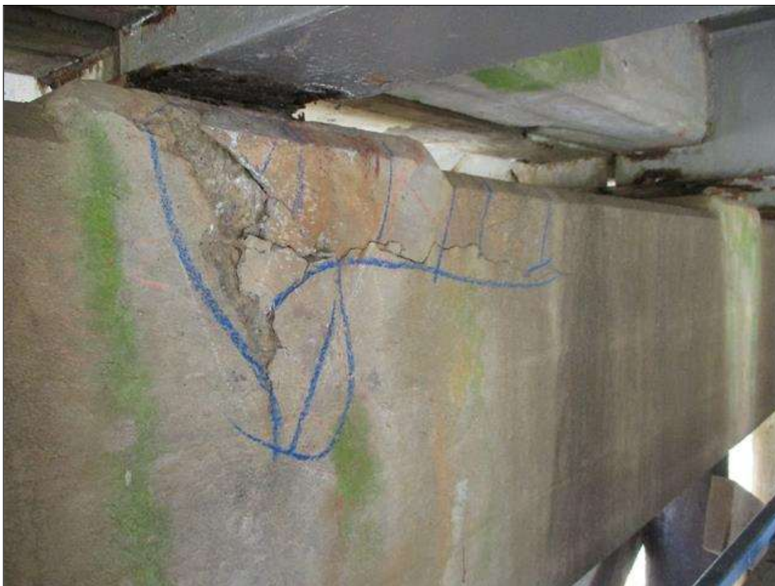
Bent 2 Cap 1: SOUTH FACE AT BEAM 2, TOP 10" OF THE CAP, APPROXIMATELY 2 SQUARE FEET OF MAP CRACKING TO 1/8" WIDE WITH ASSOCIATED DELAMINATION AND SPALLING TO 3/4" DEEP
