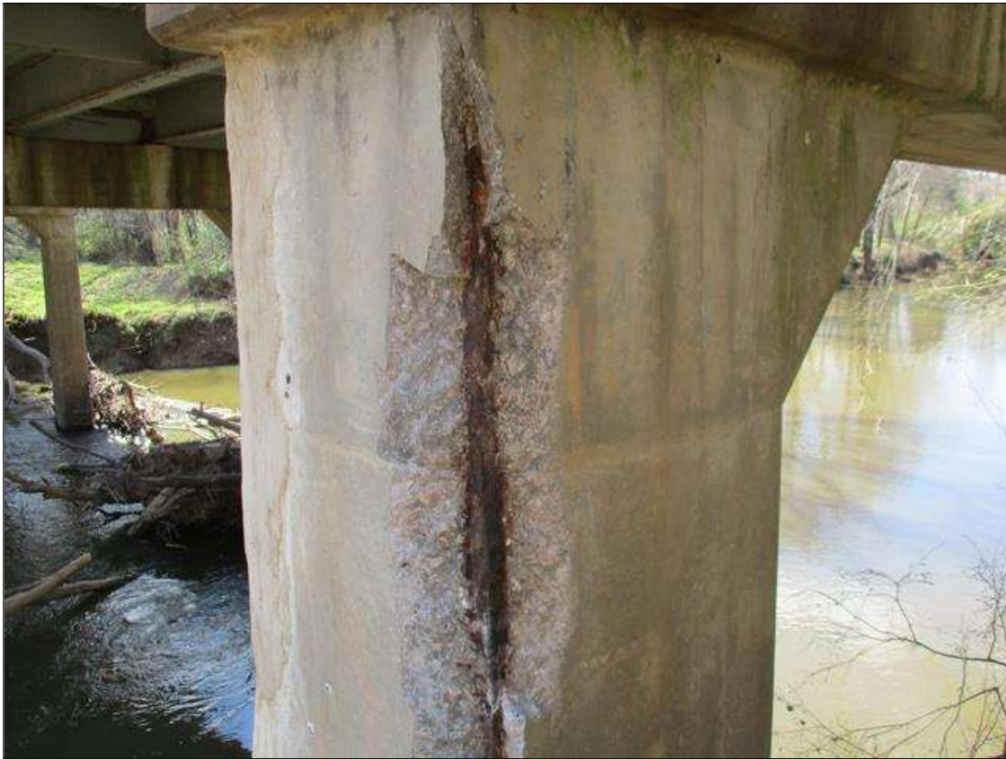
Bent 7 Pile 2: [PROMPT ACTION REQUEST] NORTHEAST CORNER, SPALLING WITH EXPOSED REBAR UP TO 2" DEEP, VERTICAL CRACKING TO 1/8" WIDE AND ASSOCIATED DELAMINATION [TOTAL AREA APPROXIMATELY 8' LONG X 1' WIDE]
