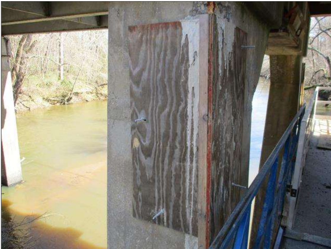
Bent 5 Pile 1: SOUND PATCHING --> [FORMERLY 2.75' X 7" X 6" DEEP SPALL WITH EXPOSED REBAR]
