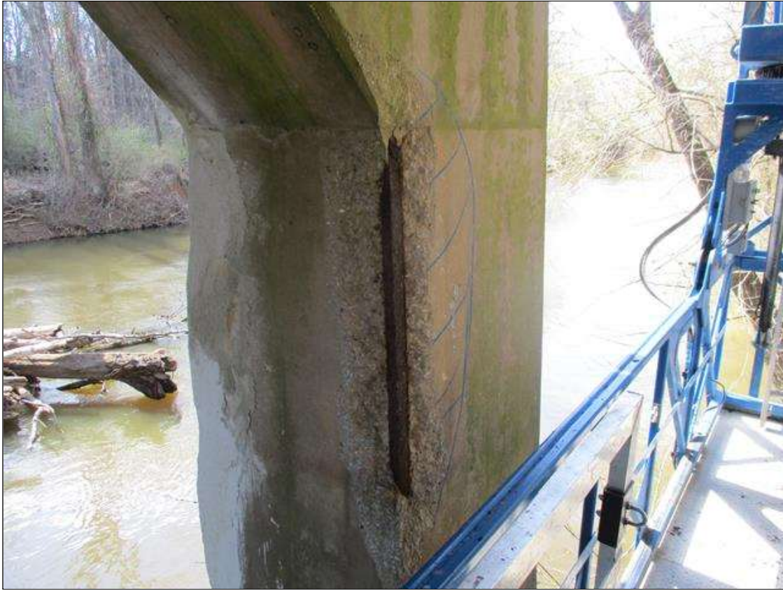
Bent 7 Pile 1: [PROMPT ACTION REQUEST] 4' X 6" X 7" SPALL WITH EXPOSED REBAR ON NORTHEAST CORNER, NO MEASURABLE SECTION LOSS, WITH APPROXIMATELY 3 SQUARE FEET ASSOCIATED DELAMINATION
