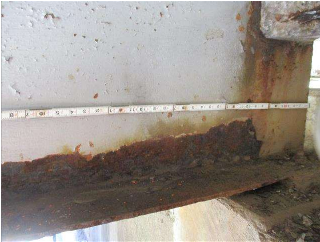
Span 8 Beam 2: [PROMPT ACTION REQUEST] 8" OUT FROM THE BEAM END AT BENT 8, IN THE LOWER 4" OF THE WEB, CORROSION WITH APPROXIMATELY 3/16" SECTION LOSS [AVERAGE 1/4" REMAINS] FOR 30" LONG.
