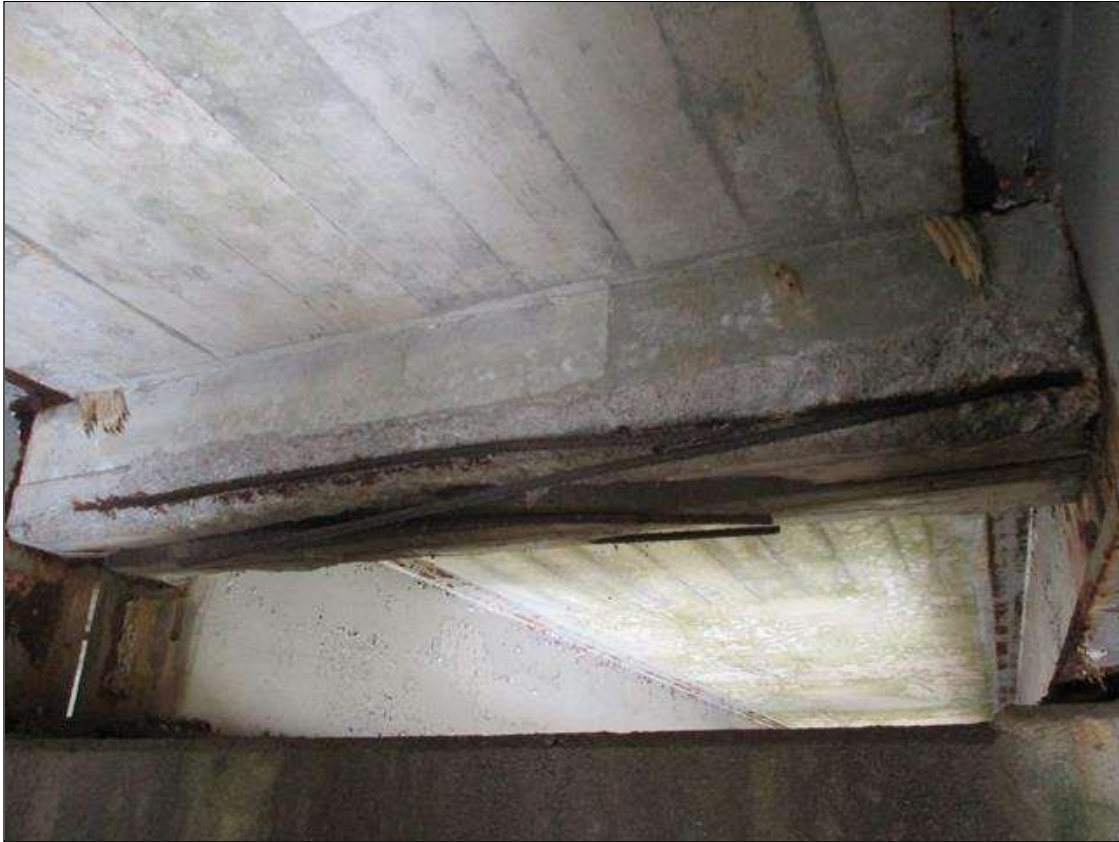
Span 5 Beam 2: [PROMPT ACTION REQUEST] BAY 2 AT BENT 5, REINFORCED CONCRETE DIAPHRAGM, SPALLING WITH EXPOSED REBAR [APPROXIMATELY 6' LONG X 12" WIDE X UP TO 3" DEEP] WITH DELAMINATED REBAR, WHICH HAS SURFACE CORROSION AND PITTING UP TO 1/8" DEEP
