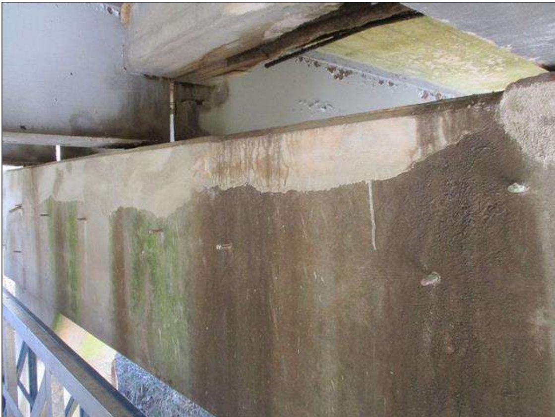
Bent 7 Cap 1: [NEW REPAIR] SOUND PATCHING - SOUTH FACE AT THE TOP OF THE CAP
