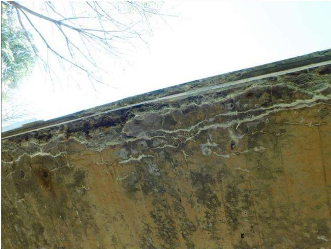
Span 1 Deck: 12' LONG X 1.5' WIDE X 4" DEEP DELAMINATION ALONG THE RIGHT SIDE OF THE SLAB BEGINNING 5' FROM THE NEAR END WITH HEAVY EFFLORESCENCE BUILDUP AND ONE LONGITUDINAL STEEL BAR EXPOSED. STEEL IS CORRODING WITH 0.0625" PITTING AND SCALE. (PAR)
