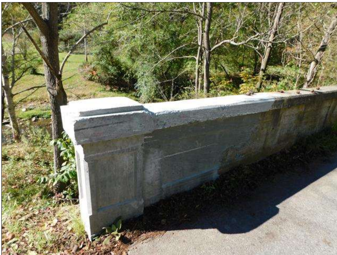
Span 1 Left Bridge Rail: NEAR END OF THE LEFT RAIL HAS BEEN RE-POURED FOR 8' LONG AS REPAIRS TO PREVIOUS PAR.
