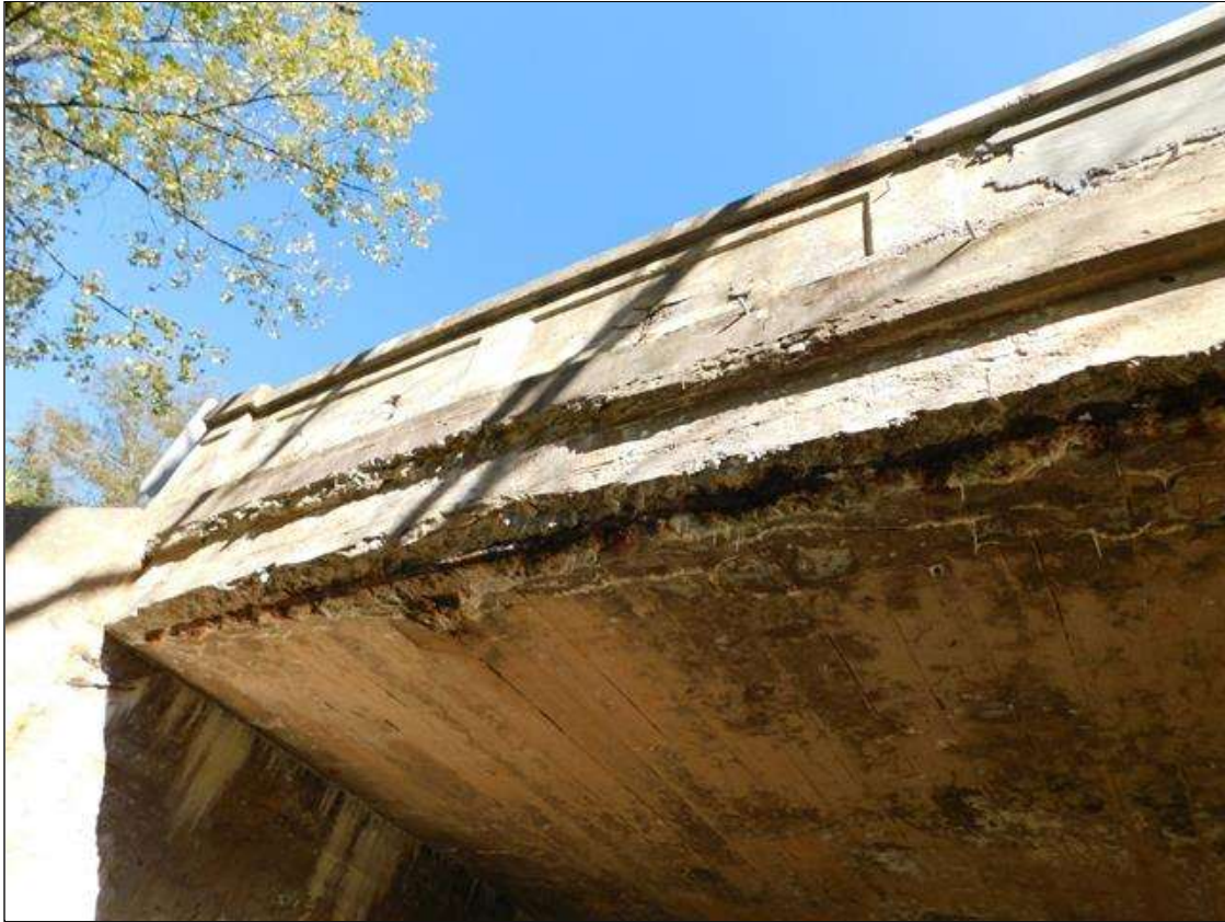
Span 1 Deck: 1.5' WIDE X FULL LENGTH X 6" DEEP DELAMINATION ALONG THE LEFT SIDE OF THE SLAB WITH HEAVY EFFLORESCENCE BUILDUP AND ONE EXPOSED LONGITUDINAL STEEL BAR. STEEL IS CORRODING WITH 0.0625" PITTING AND SCALE LOSS. (PAR)
