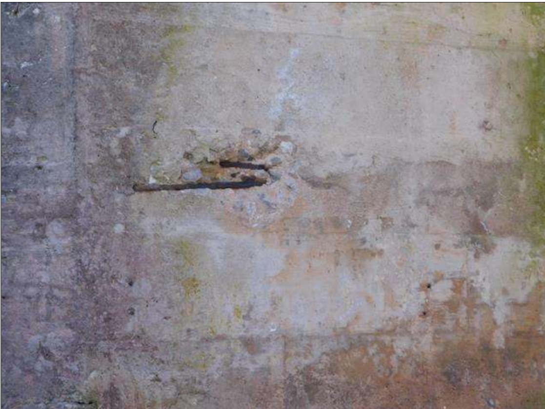
End Bent 1 Abutment: 1' WIDE X 9" HIGH X 2" DEEP DELAMINATION WITH EXPOSED AND CORRODING REINFORCING STEEL AT THE RIGHT SIDE OF THE END BENT, 5' UP FROM THE GROUND. (PAR)
