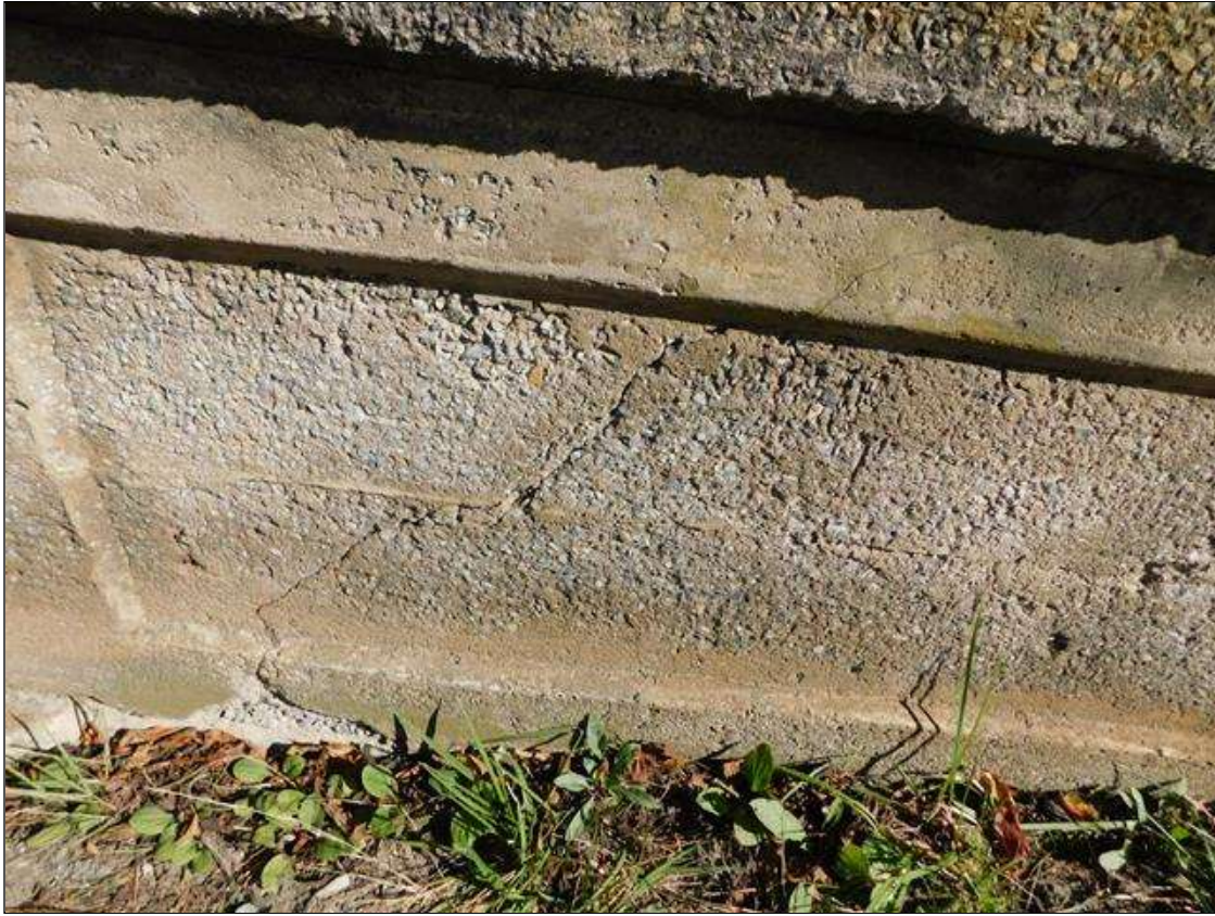
Span 1 Right Bridge Rail: 0.125" WIDE DIAGONAL CRACK BEGINNING AT 5.5' FROM THE FAR END AT THE TOP OF THE RAIL AND RUNNING BACK TOWARDS THE FAR END. SPALL AT FAR END OF RAIL HAS BEEN PATCHED AS REPAIR TO PREVIOUS PAR.
