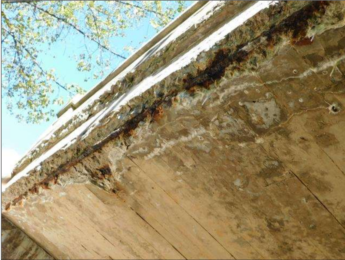
Span 1 Deck: 1.5' WIDE X FULL LENGTH X 6" DEEP DELAMINATION ALONG THE LEFT SIDE OF THE SLAB WITH HEAVY EFFLORESCENCE BUILDUP AND ONE EXPOSED LONGITUDINAL STEEL BAR. STEEL IS CORRODING WITH 0.0625" PITTING AND SCALE LOSS. (PAR)
