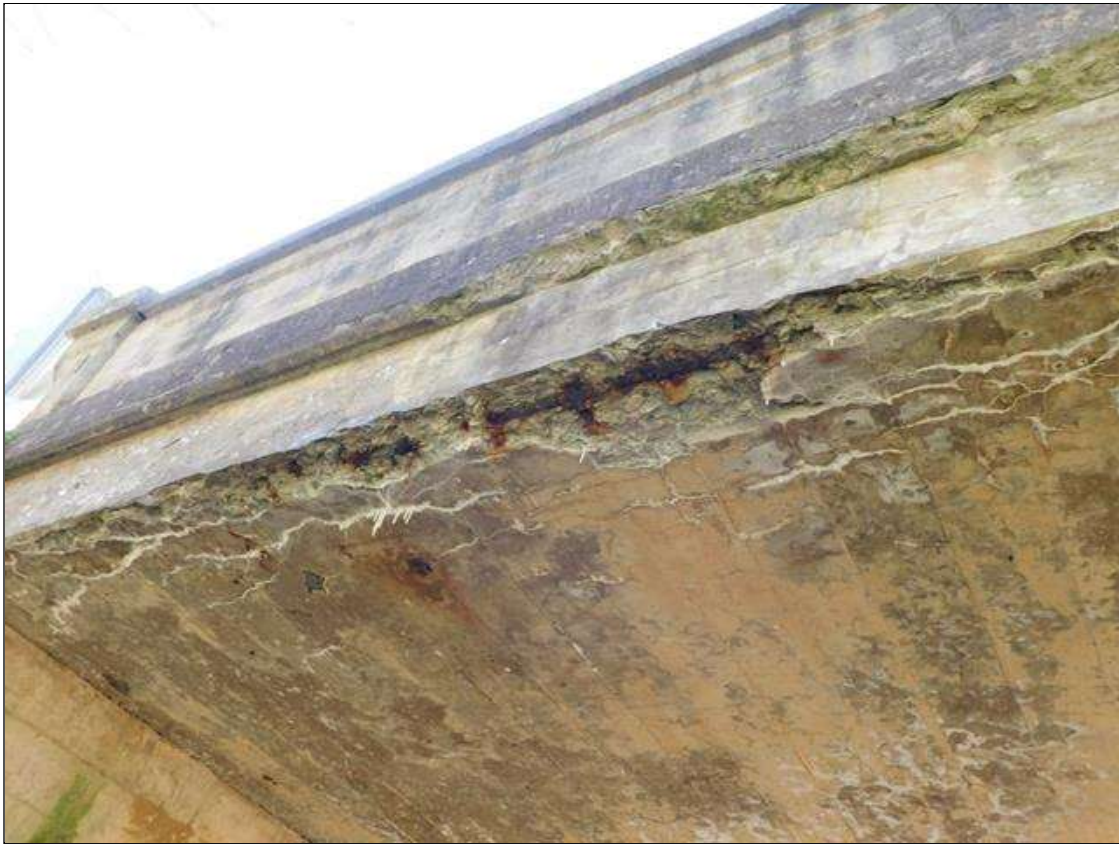
Span 1 Deck: 12' LONG X 1.5' WIDE X 4" DEEP DELAMINATION ALONG THE RIGHT SIDE OF THE SLAB BEGINNING 5' FROM THE NEAR END WITH HEAVY EFFLORESCENCE BUILDUP AND ONE LONGITUDINAL STEEL BAR EXPOSED. STEEL IS CORRODING WITH 0.0625" PITTING AND SCALE. (PAR)
