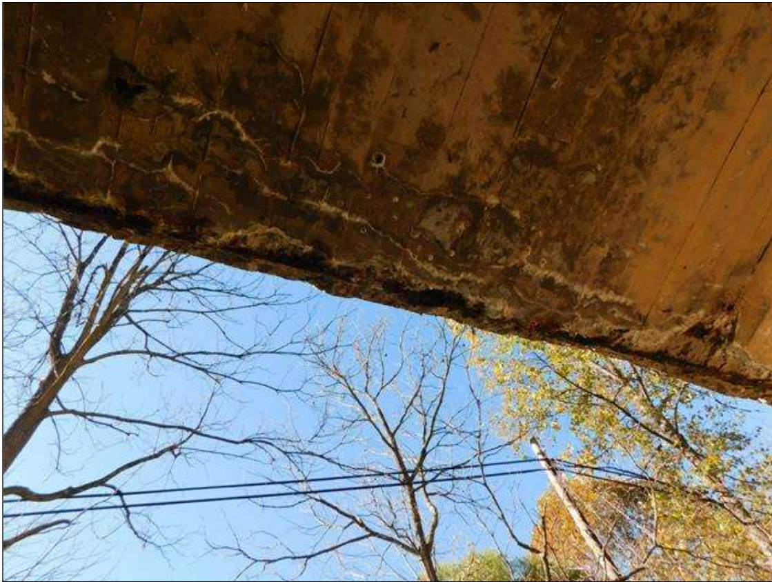
Span 1 Deck: 1.5' WIDE X FULL LENGTH X 6" DEEP DELAMINATION ALONG THE LEFT SIDE OF THE SLAB WITH HEAVY EFFLORESCENCE BUILDUP AND ONE EXPOSED LONGITUDINAL STEEL BAR. STEEL IS CORRODING WITH 0.0625" PITTING AND SCALE LOSS. (PAR)
