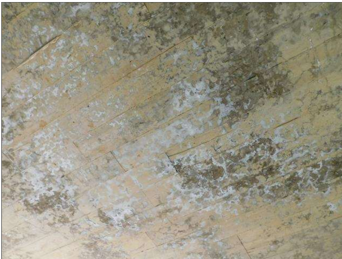
Span 1 Deck: HAIRLINE MAP CRACKS SCATTERED THROUGHOUT THE UNDERSIDE OF THE SLAB.
