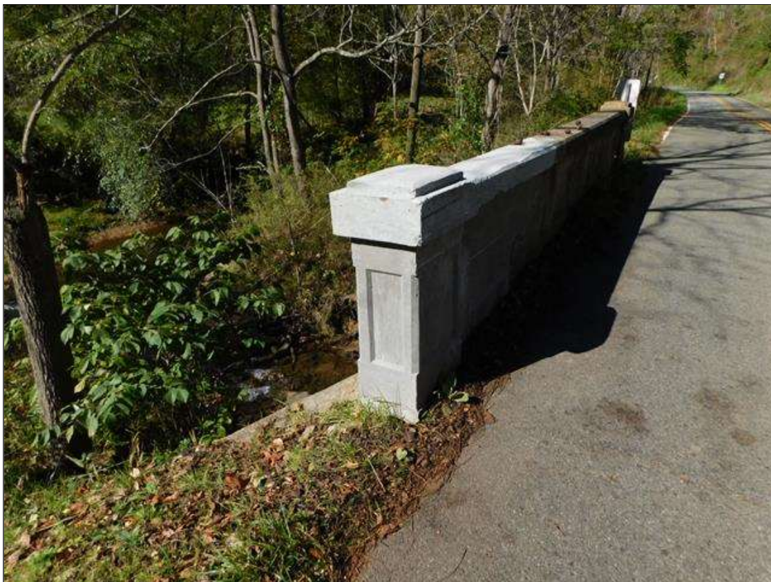
DELINEATOR AT SOUTH WEST CORNER MISSING. (PAR)
