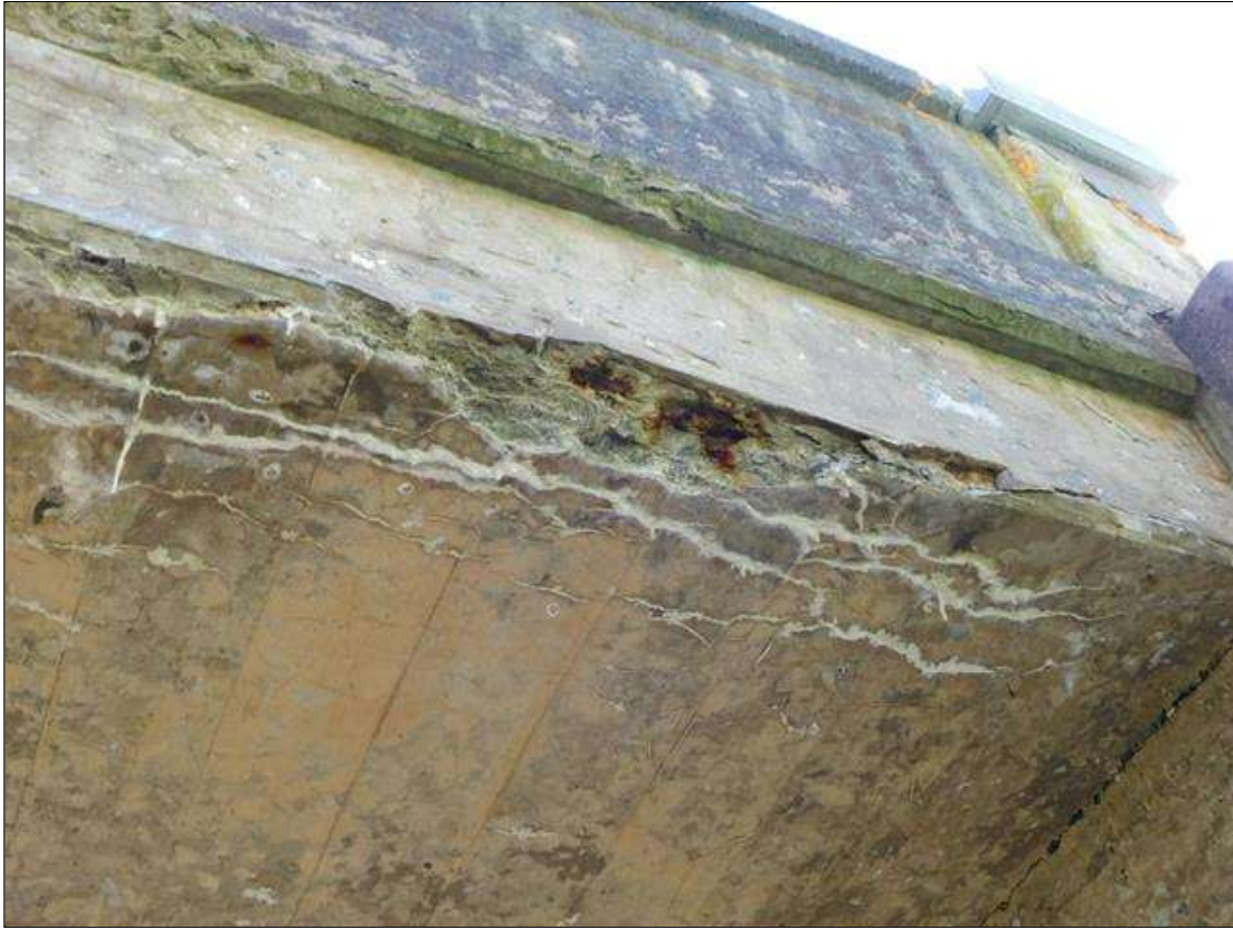
Span 1 Deck: 12' LONG X 1.5' WIDE X 4" DEEP DELAMINATION ALONG THE RIGHT SIDE OF THE SLAB BEGINNING 5' FROM THE NEAR END WITH HEAVY EFFLORESCENCE BUILDUP AND ONE LONGITUDINAL STEEL BAR EXPOSED. STEEL IS CORRODING WITH 0.0625" PITTING AND SCALE. (PAR)
