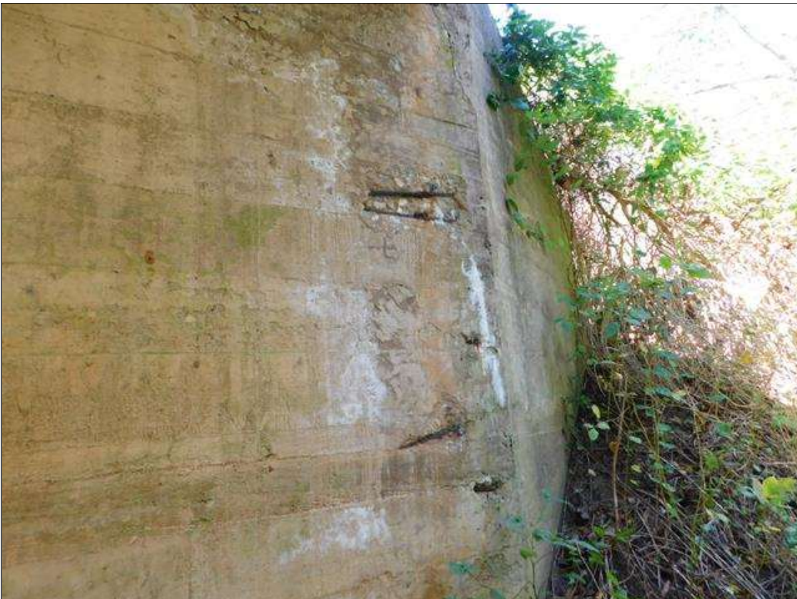
End Bent 2 Abutment: MULTIPLE SPALLS UP TO 2' WIDE X 6" HIGH ALONG THE RIGHT SIDE OF THE END BENT WITH REINFORCING STEEL EXPOSED AND CORRODING. (PAR)
