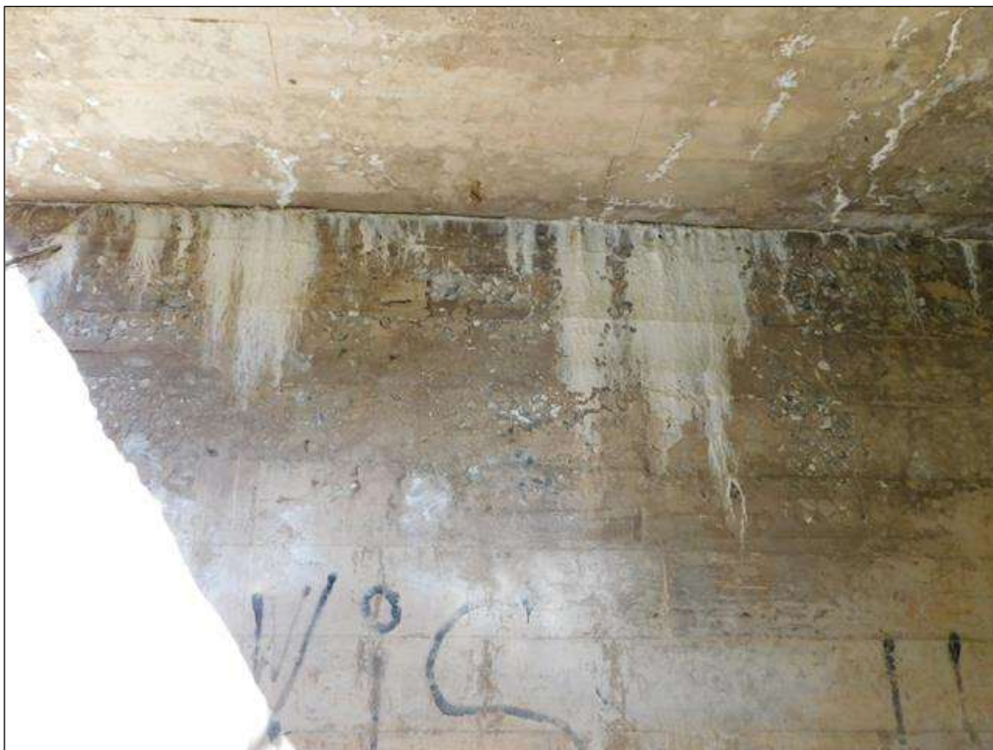
End Bent 1 Abutment: EFFLORESCENCE BUILDUP EMANATING FROM BRIDGE SEAT.
