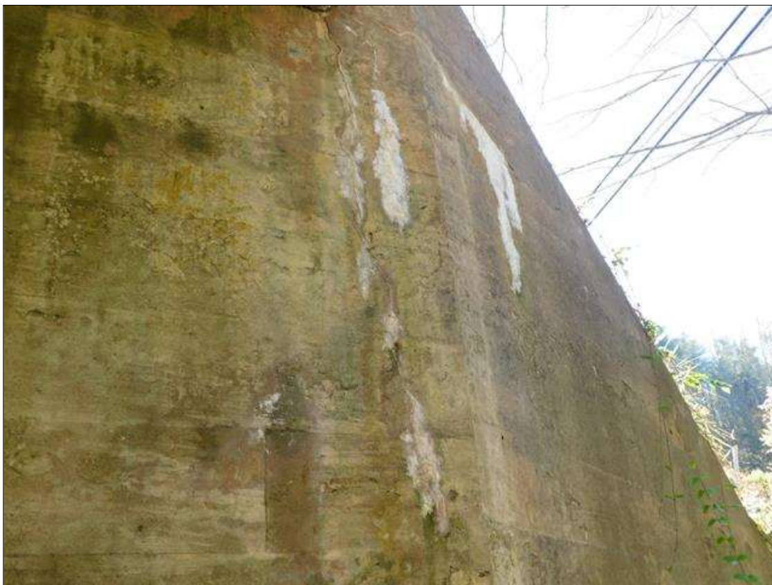
End Bent 1 Abutment: DIAGONAL CRACKS WITH EFFLORESCENCE IN LEFT END NEAR BREAKBACK.
