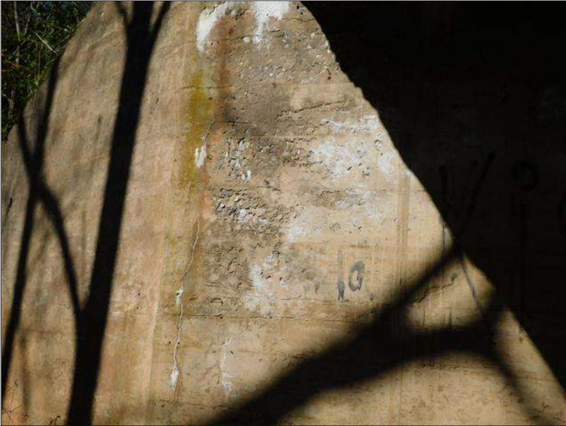
End Bent 2 Abutment: HEAVY EFFLORESCENCE BUILDUP ALONG THE BRIDGE SEAT AND RANDOM HAIRLINE CRACKS WITH EFFLORESCENCE STAINING
