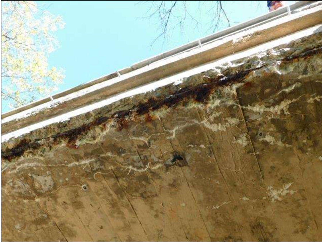
Span 1 Deck: 1.5' WIDE X FULL LENGTH X 6" DEEP DELAMINATION ALONG THE LEFT SIDE OF THE SLAB WITH HEAVY EFFLORESCENCE BUILDUP AND ONE EXPOSED LONGITUDINAL STEEL BAR. STEEL IS CORRODING WITH 0.0625" PITTING AND SCALE LOSS. (PAR)
