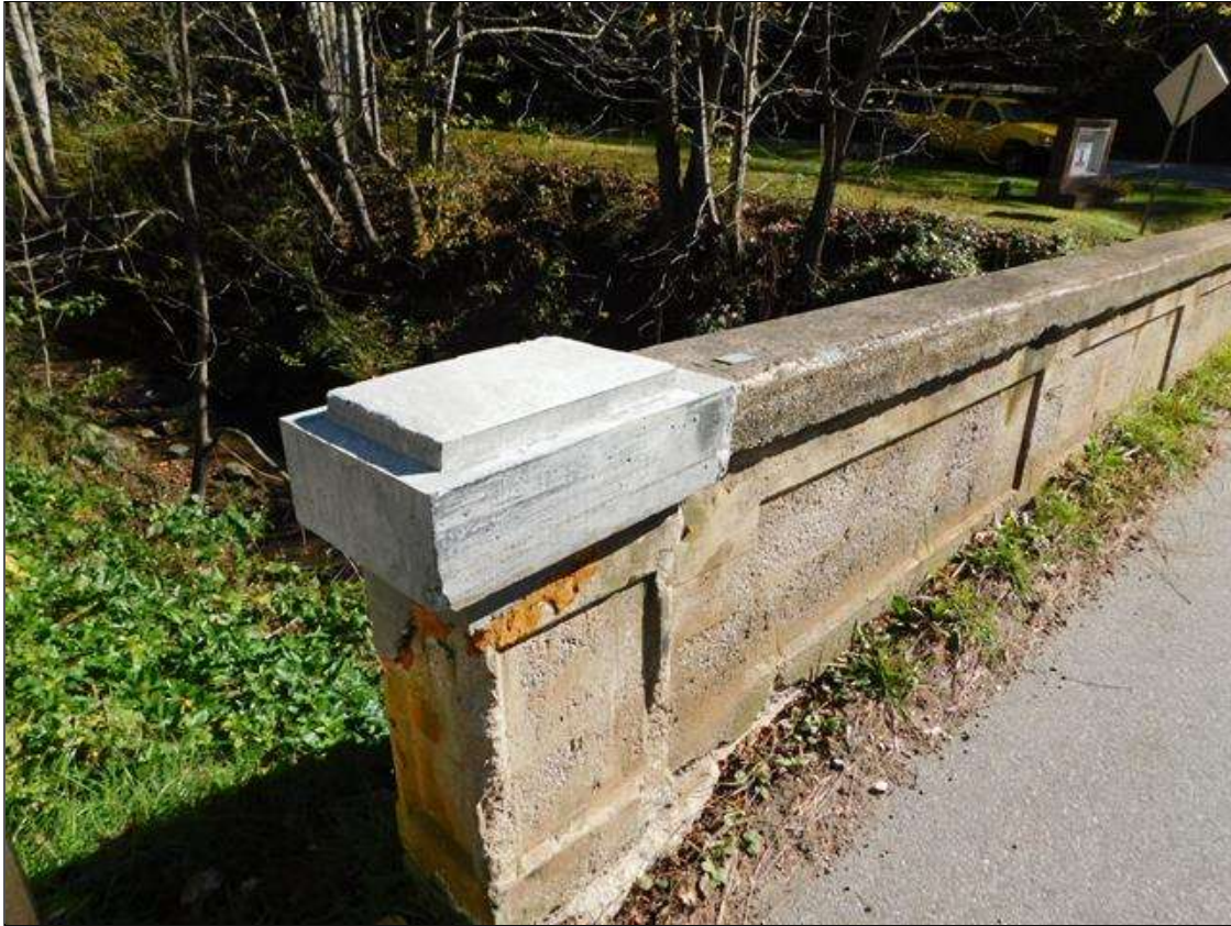
Span 1 Right Bridge Rail: 0.125" WIDE DIAGONAL CRACK BEGINNING AT 5.5' FROM THE FAR END AT THE TOP OF THE RAIL AND RUNNING BACK TOWARDS THE FAR END. SPALL AT FAR END OF RAIL HAS BEEN PATCHED AS REPAIR TO PREVIOUS PAR.
