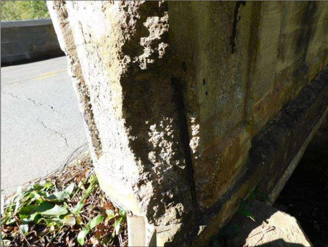
Span 1 Right Bridge Rail: 9" WIDE X 1.5' HIGH X 4" DEEP SPALL IN NEAR END WITH ONE VERTICAL BAR EXPOSED AND CORRODING. (PAR)
