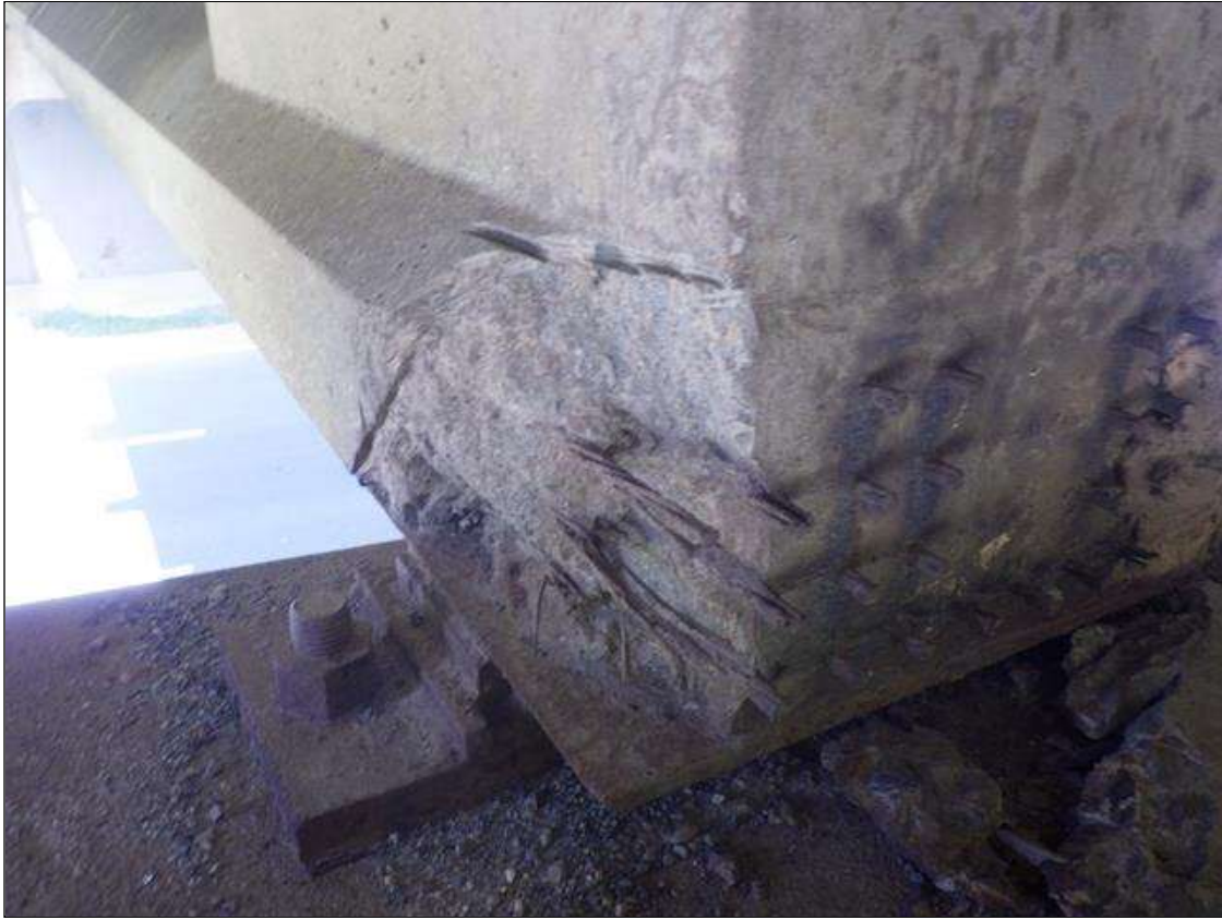
Span 2 Beam 4: 1 FOOT 4 INCHES LONG X 10 INCHES HIGH X 4 INCHES WIDE SPALLED AREA WITH (5) EXPOSED PRESTRESSING STRANDS IN THE RIGHT BOTTOM FLANGE AT BENT 2 (PRIORITY ACTION REQUEST)
