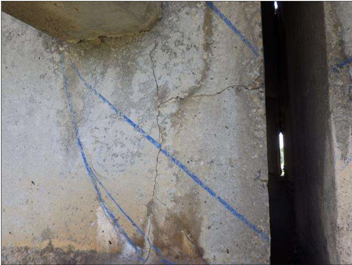
Span 3 Beam 1: DELAMINATED AREA UP TO 1 FOOT 3 INCHES LONG X FULL HEIGHT X FULL WIDTH IN THE LEFT SIDE OF WEB AT BENT 2
