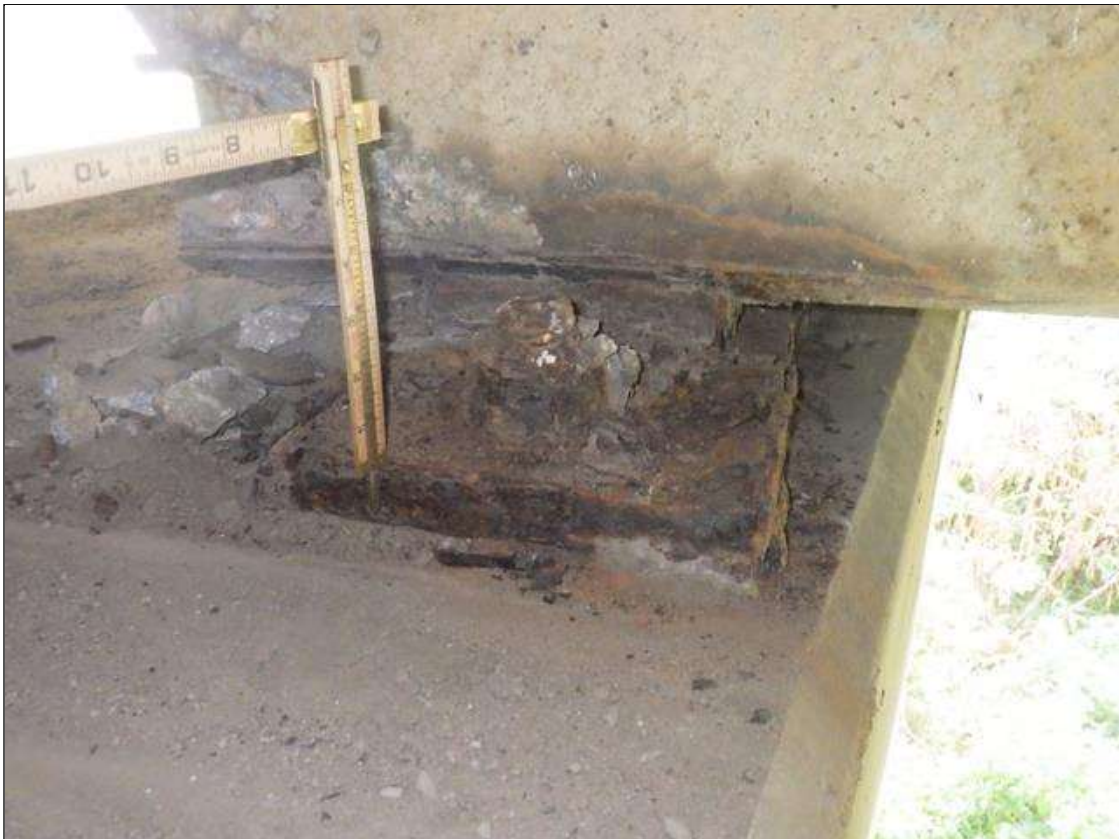
Span 1 Beam 2 - Far Bearing: ACTIVE CORROSION UP TO FULL PERIMETER X FULL HEIGHT WITH 1/32 INCH SECTION LOSS THROUGHOUT GIRDER 2 BEARING
