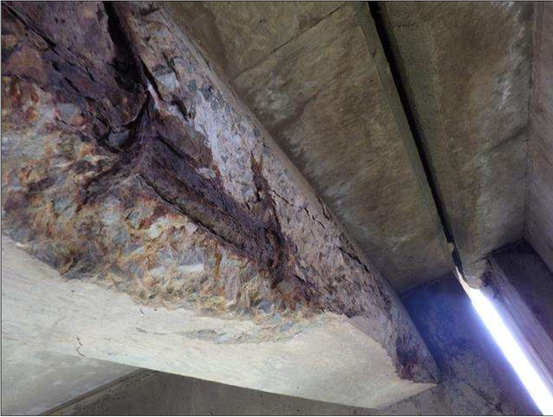
Span 3 Beam 3: SPALLED AREA UP TO FULL LENGTH X 6 INCHES WIDE X FULL HEIGHT WITH EXPOSED REINFORCEMENT IN BAY 3 END DIAPHRAGM AT BENT 2
