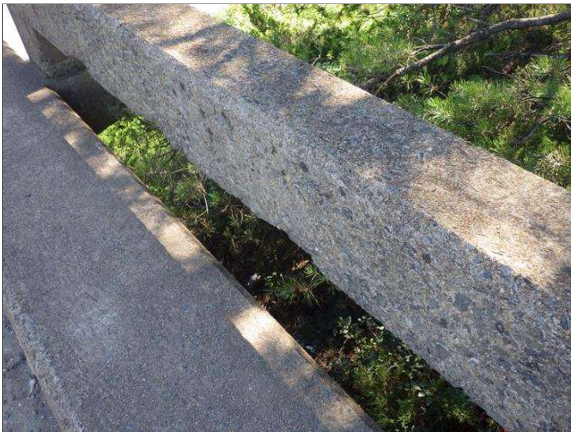
Span 4 Left Bridge Rail: INTERMITTENT 3 FEET 6 INCHES LONG X 3 INCHES HIGH X 1 INCH WIDE SPALLED AREA IN THE RAIL BETWEEN POST 3 AND POST 4
