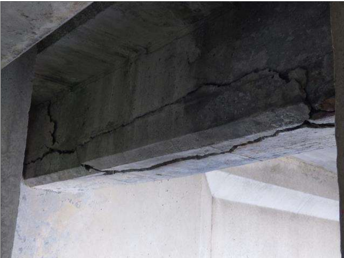
Span 2 Beam 2: DELAMINATED UP TO FULL LENGTH X FULL WIDTH X FULL HEIGHT IN BAY 2 END DIAPHRAGM AT BENT 1
