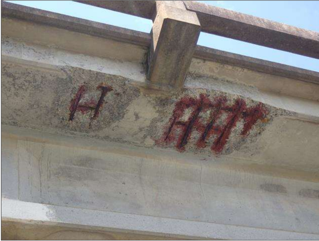
Span 2 Deck: INTERMITTENT 10 FEET LONG X 2 FEET 6 INCHES WIDE X 6 INCHES HIGH SPALLED AREA WITH EXPOSED REINFORCEMENT (10 PERCENT SECTION LOSS TO REBAR) IN THE UNDERSIDE OF THE SOUTH OVERHANG, 7 FEET FROM BENT 1 AND ABOVE THE MERGE LANE (PRIORITY ACTION REQUEST)
