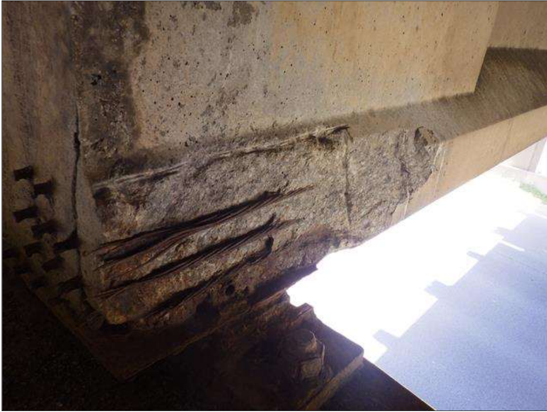
Span 2 Beam 3: 2 FOOT 8 INCHES LONG X 10 INCHES HIGH X 4 INCHES WIDE SPALLED AREA WITH (3) EXPOSED PRESTRESSING STRANDS IN THE LEFT BOTTOM FLANGE AT BENT 2 (PRIORITY ACTION REQUEST)
