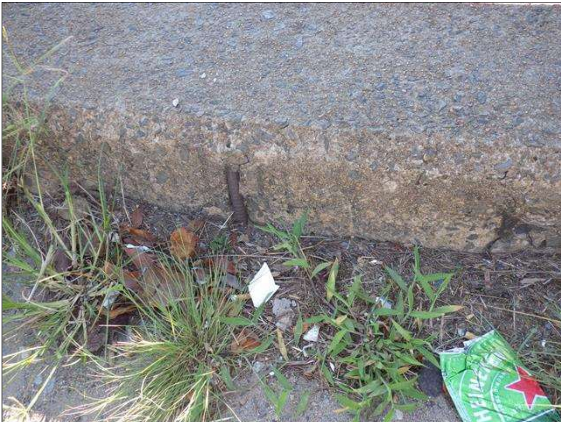
Span 1 Right Bridge Rail: (4) SPALLED AREAS UP TO 6 INCHES HIGH X 2 INCHES LONG X 1/2 INCH DEEP WITH EXPOSED REINFORCEMENT IN THE CURB
