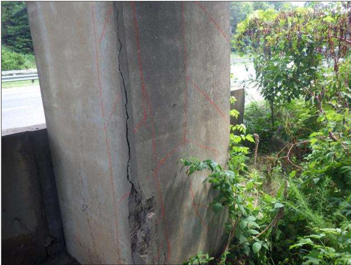
Bent 1 Pile 2: DELAMINATED AND SPALLED AREA UP TO FULL HEIGHT X FULL LENGTH X 1 FOOT 2 INCHES WIDE IN THE WEST, NORTH, AND SOUTH FACES
