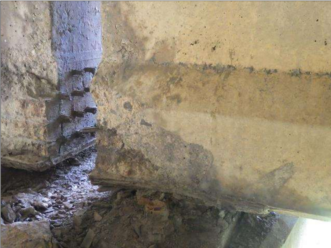
Span 1 Beam 4: 1 FOOT LONG X 9 INCHES HIGH X 2 INCHES WIDE SPALLED AREA WITH (2) EXPOSED PRESTRESSING STRANDS IN THE LEFT BOTTOM FLANGE AT BENT 1 (PRIORITY ACTION REQUEST)
