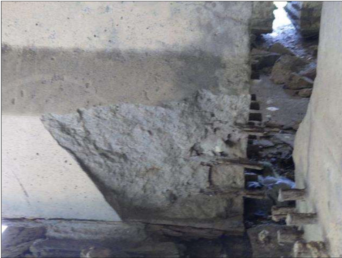
Span 2 Beam 4: 1 FOOT LONG X 10 INCHES HIGH X 2 INCHES WIDE SPALLED AREA WITH (3) EXPOSED PRESTRESSING STRANDS IN THE LEFT BOTTOM FLANGE AT BENT 1 (PRIORITY ACTION REQUEST)
