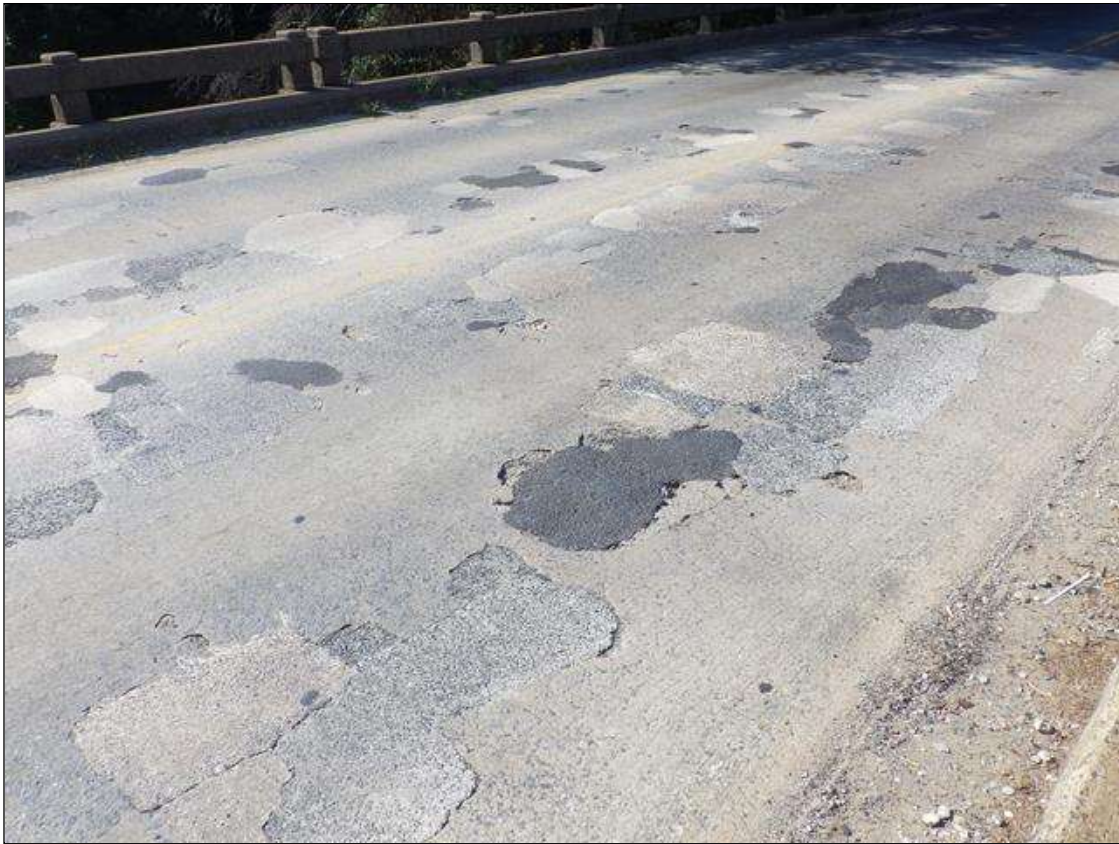
Span 1 Deck: INTERMITTENT FULL LENGTH X INTERMITTENT FULL WIDTH X UP TO 1 1/2 INCHES DEEP DELAMINATIONS, SPALLS, AND FAILED PATCHES THROUGHOUT THE DECK WITH 30 PERCENT OF DECK AREA AFFECTED
