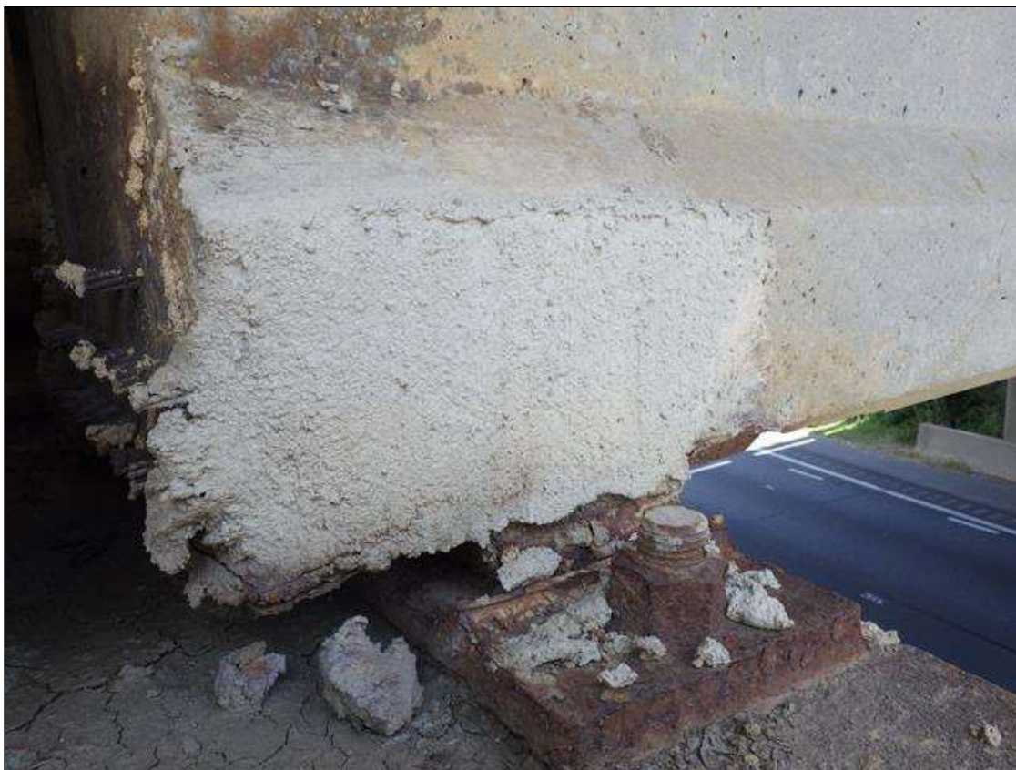
Span 3 Beam 4: PATCHED AREA UP TO 1 FOOT 4 INCHES LONG X 10 INCHES HIGH X 3 INCHES WIDE IN THE RIGHT BOTTOM FLANGE AT BENT 2
