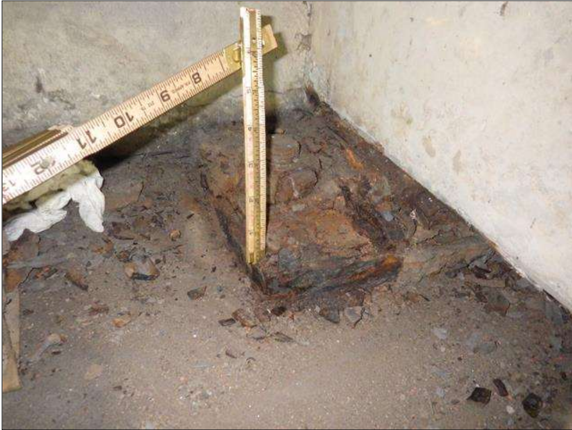
Span 1 Beam 1 - Near Bearing: ACTIVE CORROSION UP TO FULL PERIMETER X FULL HEIGHT WITH 1 1/4 INCHES REMAINING (GREATER THAN OR EQUAL TO 1/16 INCH SECTION LOSS AND LESS THAN 25 PERCENT SECTION LOSS) THROUGHOUT GIRDER 1 BEARING
