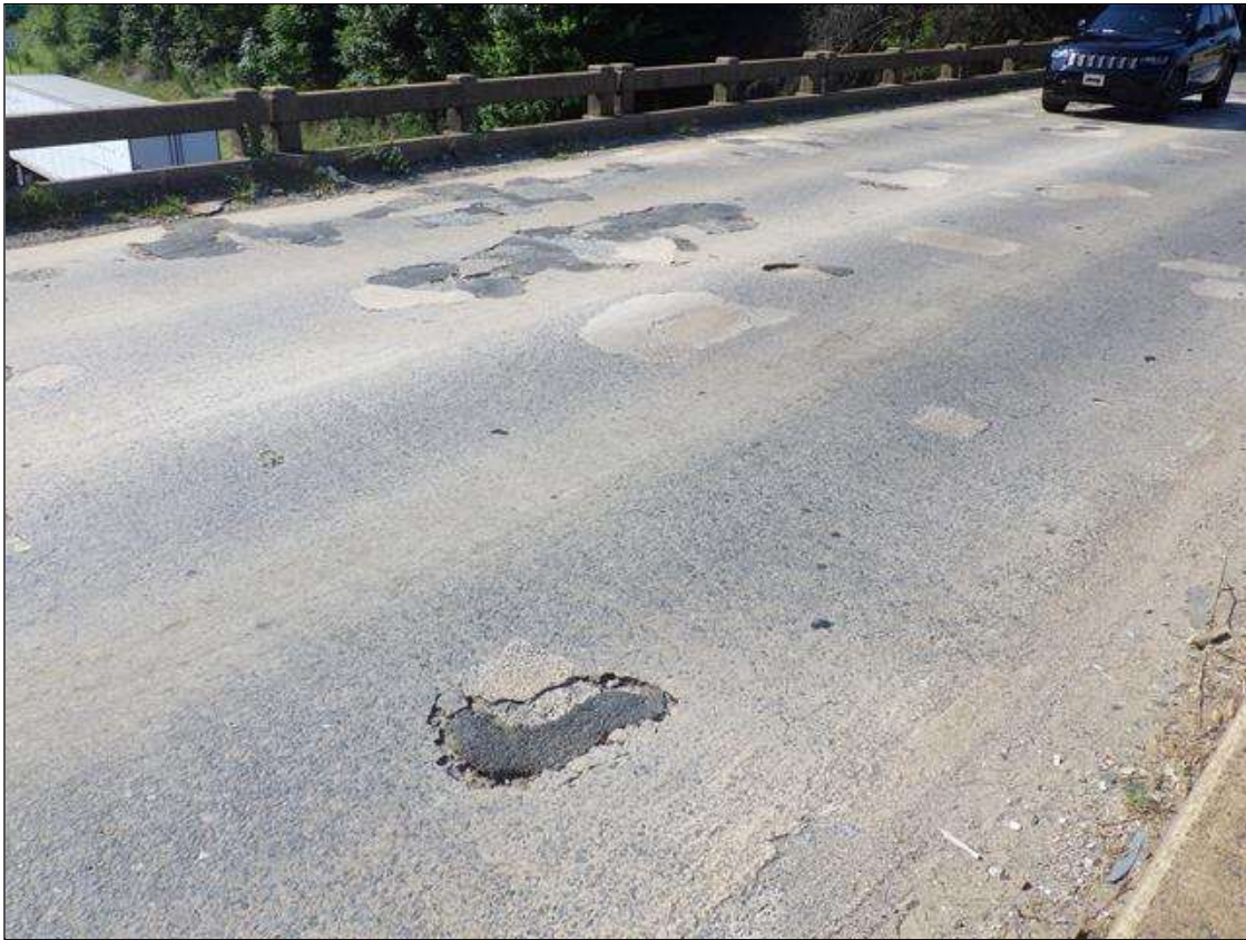
Span 2 Deck: INTERMITTENT FULL LENGTH X INTERMITTENT FULL WIDTH X UP TO 1 1/2 INCHES DEEP DELAMINATIONS, SPALLS, AND FAILED PATCHES THROUGHOUT THE DECK WITH 30 PERCENT OF DECK AREA AFFECTED
