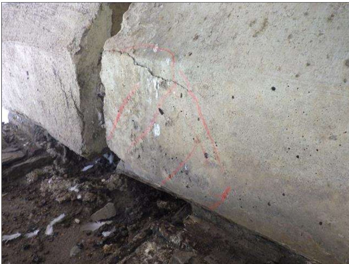
Span 4 Beam 3: DELAMINATED AREA UP TO 8 INCHES LONG X 8 INCHES HIGH IN THE RIGHT BOTTOM FLANGE AT BENT 3
