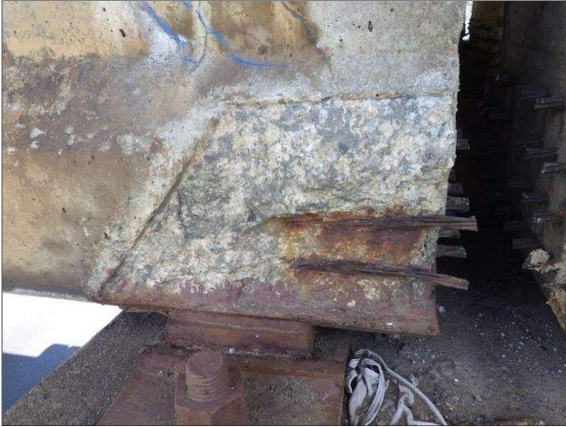
Span 3 Beam 1: 1 FOOT 2 INCHES LONG X 10 INCHES HIGH X 3 INCHES WIDE SPALLED AREA WITH (2) EXPOSED PRESTRESSING STRANDS IN THE LEFT BOTTOM FLANGE AT BENT 2 (PRIORITY ACTION REQUEST)
