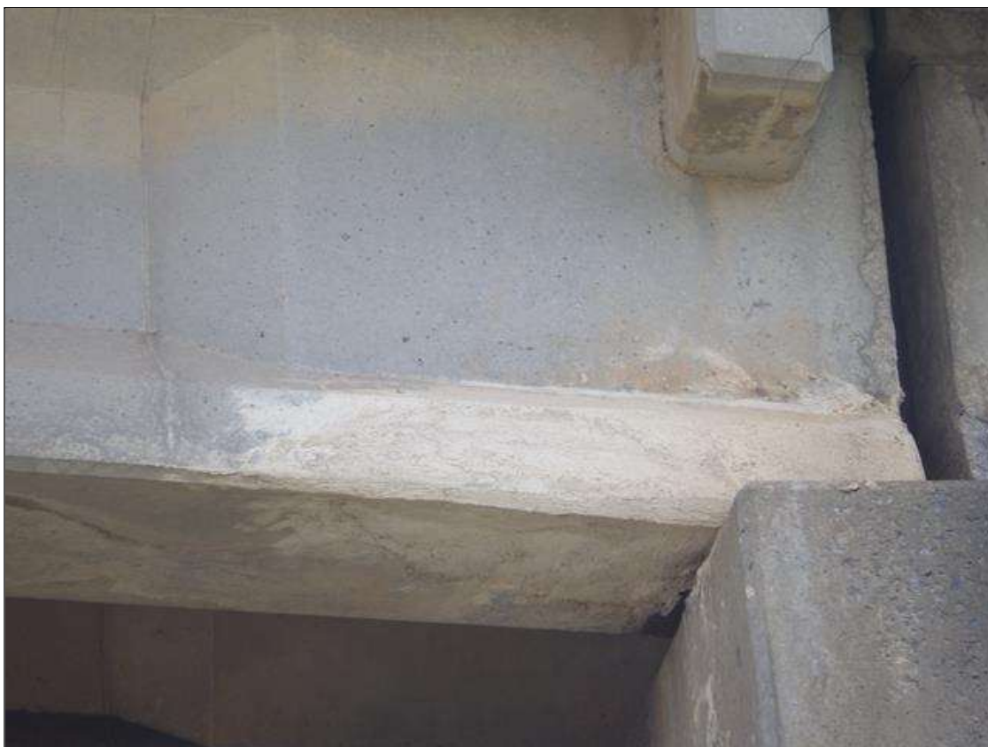
Span 2 Beam 1: PATCHED AREA UP TO 3 FEET 6 INCHES LONG X 11 INCHES HIGH X 4 INCHES WIDE IN THE LEFT BOTTOM FLANGE AT BENT 1
