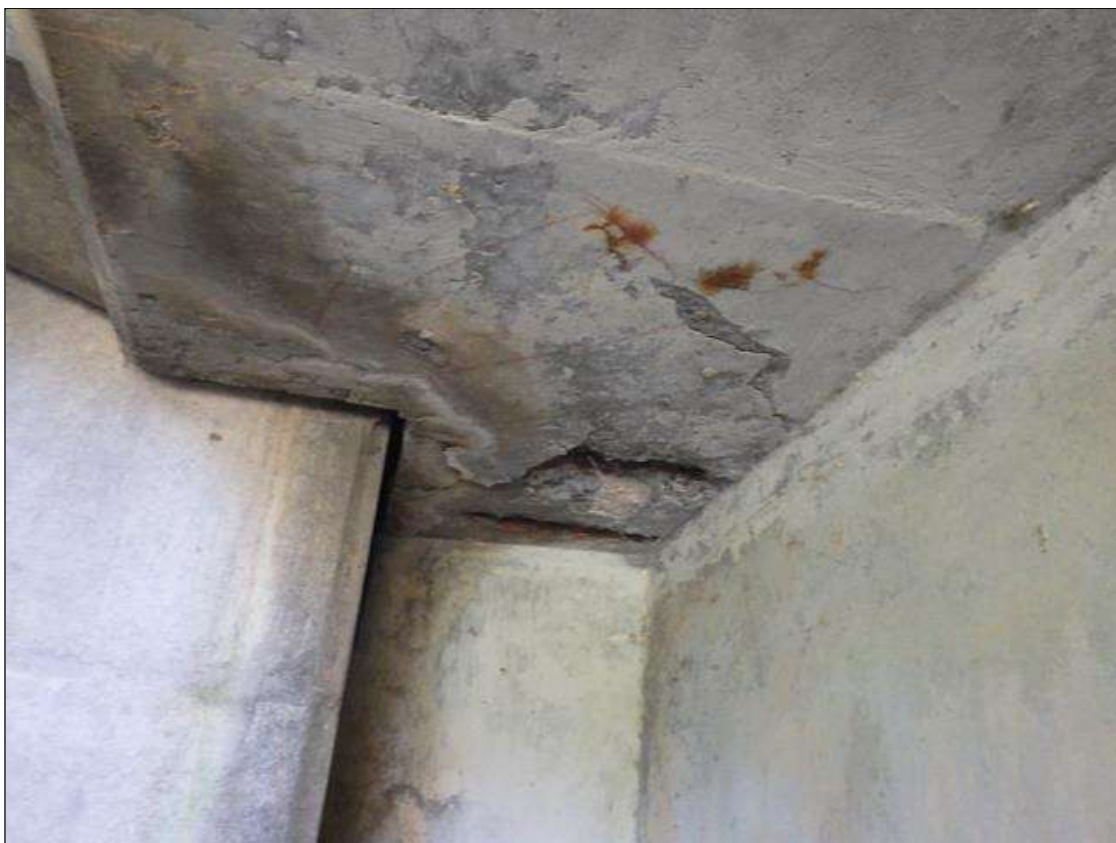
Span 1 Deck: DELAMINATED AND SPALLED AREA UP TO 2 FEET LONG X 2 FEET WIDE X 2 INCHES DEEP WITH EXPOSED REINFORCEMENT IN THE UNDERSIDE OF THE SOUTH OVERHANG AT END BENT 1
