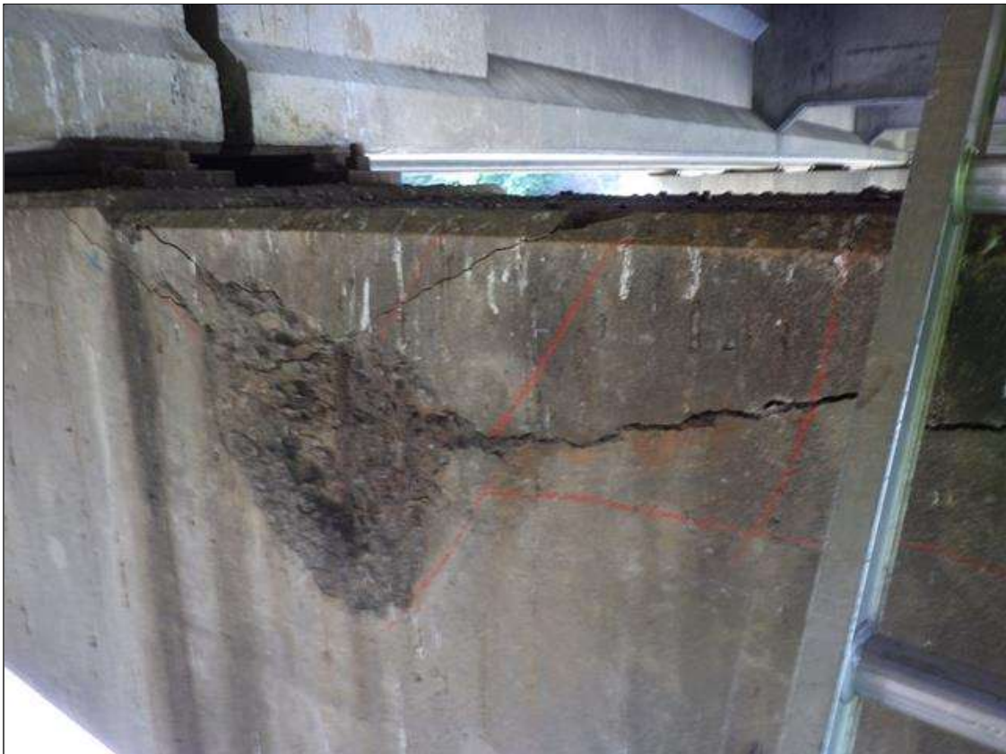
Bent 3 Cap 1: DELAMINATED AND SPALLED AREA UP TO 6 FEET X 1 FOOT 8 INCHES HIGH X 1 FOOT WIDE X 2 INCHES DEEP IN THE EAST FACE AND TOP FACE BELOW BAY 1
