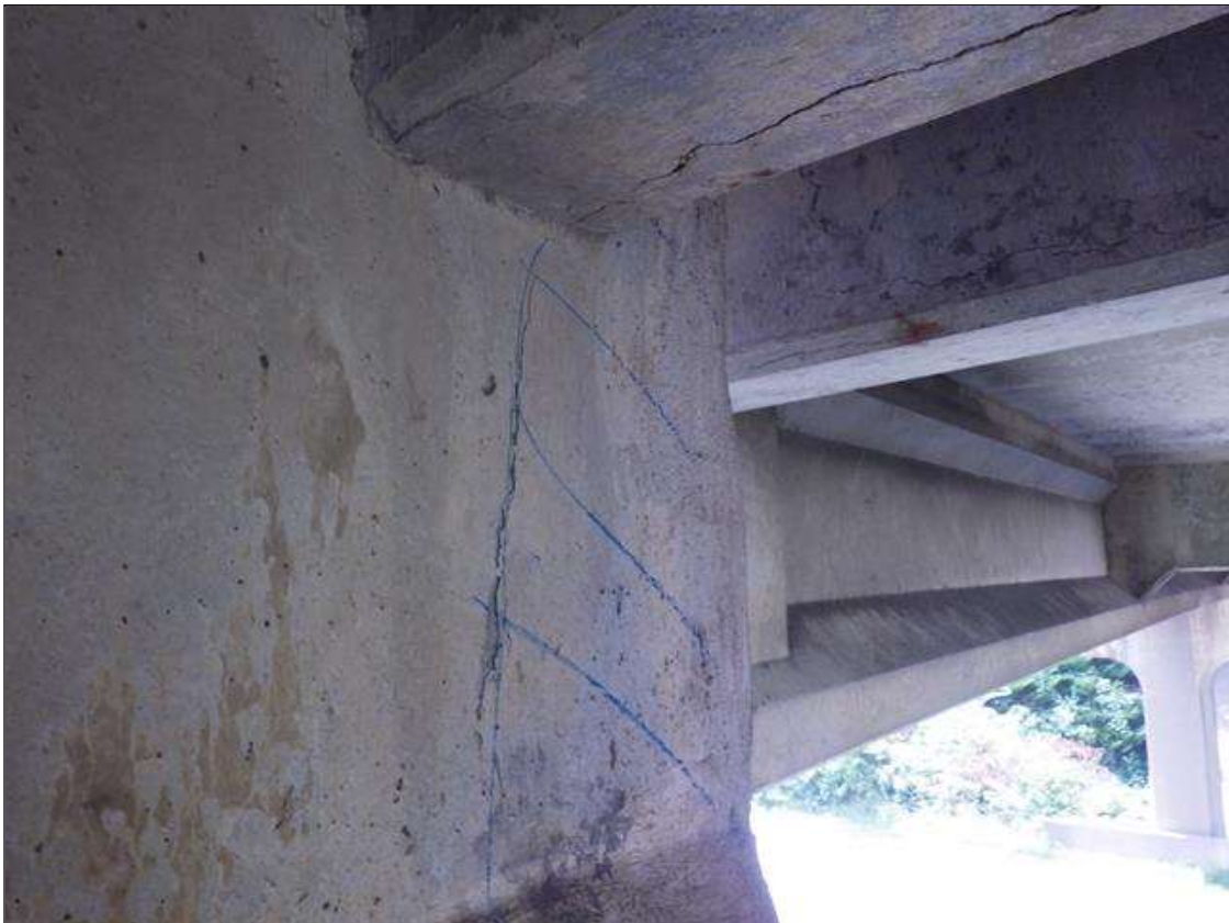
Span 3 Beam 3: DELAMINATED AREA UP TO 1 FOOT 4 INCHES LONG X FULL HEIGHT IN THE LEFT FACE OF THE WEB AT BENT 2
