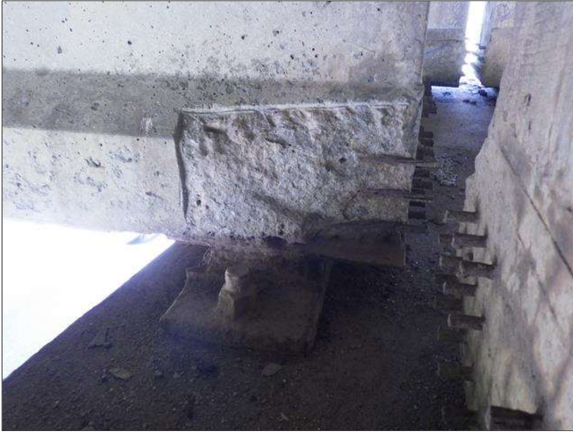
Span 2 Beam 2: 1 FOOT 2 INCHES LONG X 9 INCHES HIGH X 3 INCHES WIDE SPALLED AREA WITH (3) EXPOSED PRESTRESSING STRANDS IN THE RIGHT BOTTOM FLANGE AT BENT 2 (PRIORITY ACTION REQUEST)
