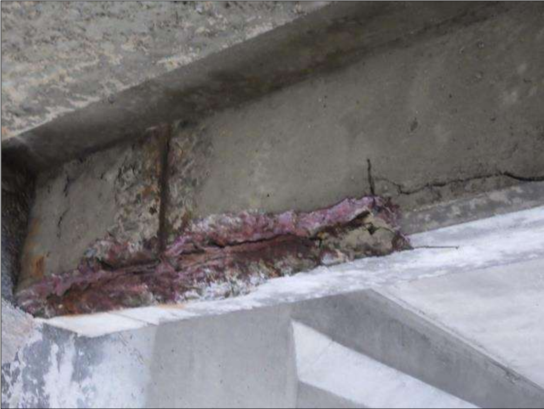
Span 3 Beam 3: DELAMINATED AND SPALLED AREA UP TO 5 FEET LONG X FULL HEIGHT X 5 INCHES WIDE WITH EXPOSED REINFORCEMENT IN BAY 3 END DIAPHRAGM AT BENT 3
