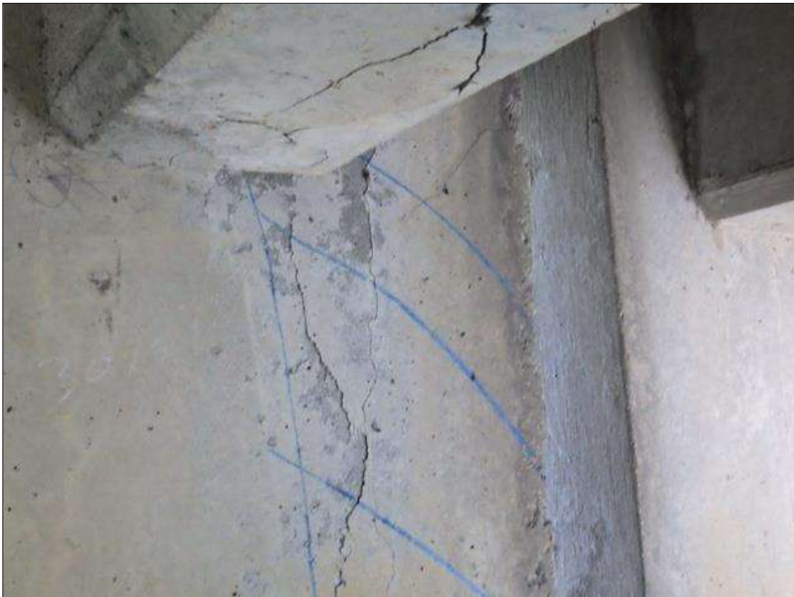
Span 1 Beam 1: DELAMINATED AREA UP TO 1 FOOT LONG X FULL HEIGHT IN THE RIGHT FACE OF THE WEB AT BENT 1
