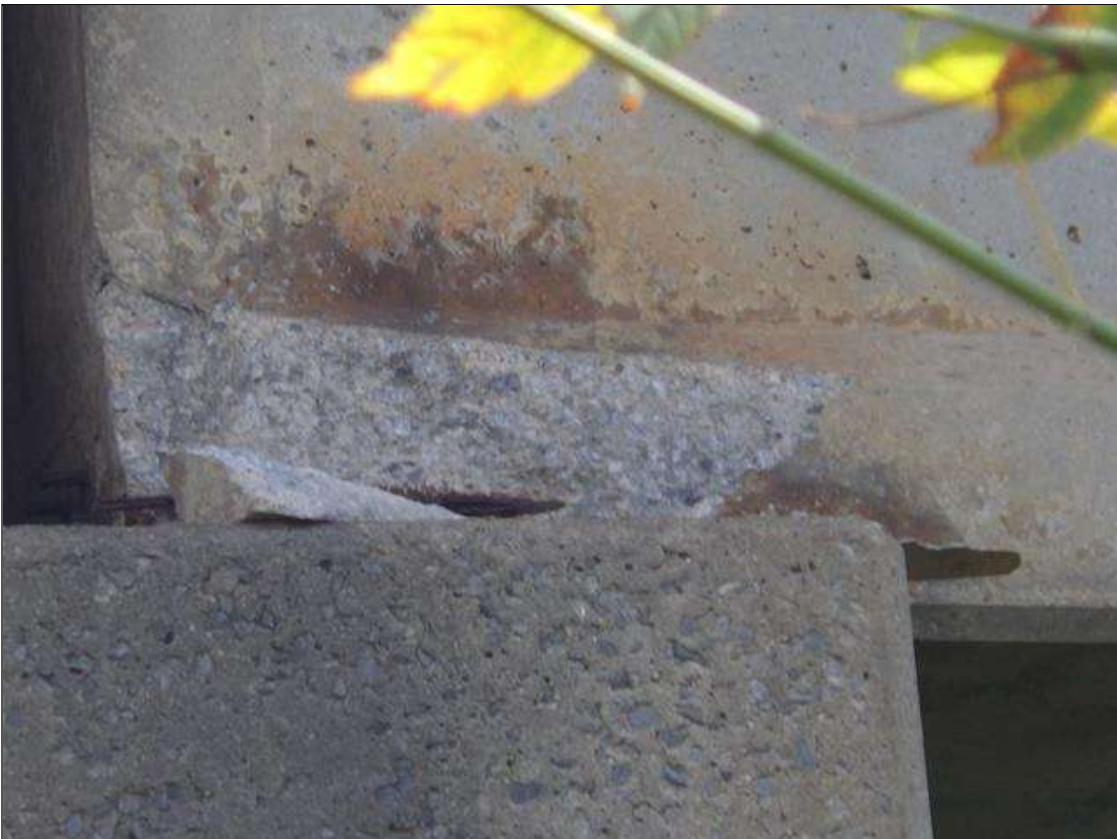
Span 1 Beam 1: 1 FOOT 8 INCHES LONG X 10 INCHES HIGH X 4 INCHES WIDE SPALLED AREA WITH (1) EXPOSED PRESTRESSING STRAND IN THE LEFT BOTTOM FLANGE AT BENT 1 (PRIORITY ACTION REQUEST)
