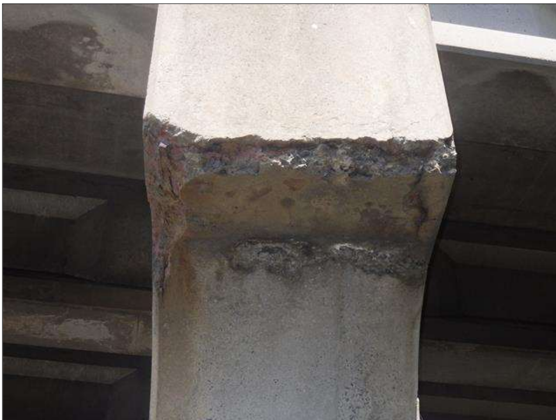
Bent 3 Cap 1: 2 FEET LONG X 3 FEET 3 INCHES WIDE X 2 INCHES HIGH SPALLED AREA WITH EXPOSED MAIN REINFORCEMENT IN THE UNDERSIDE OF THE SOUTH OVERHANG (PRIORITY ACTION REQUEST)
