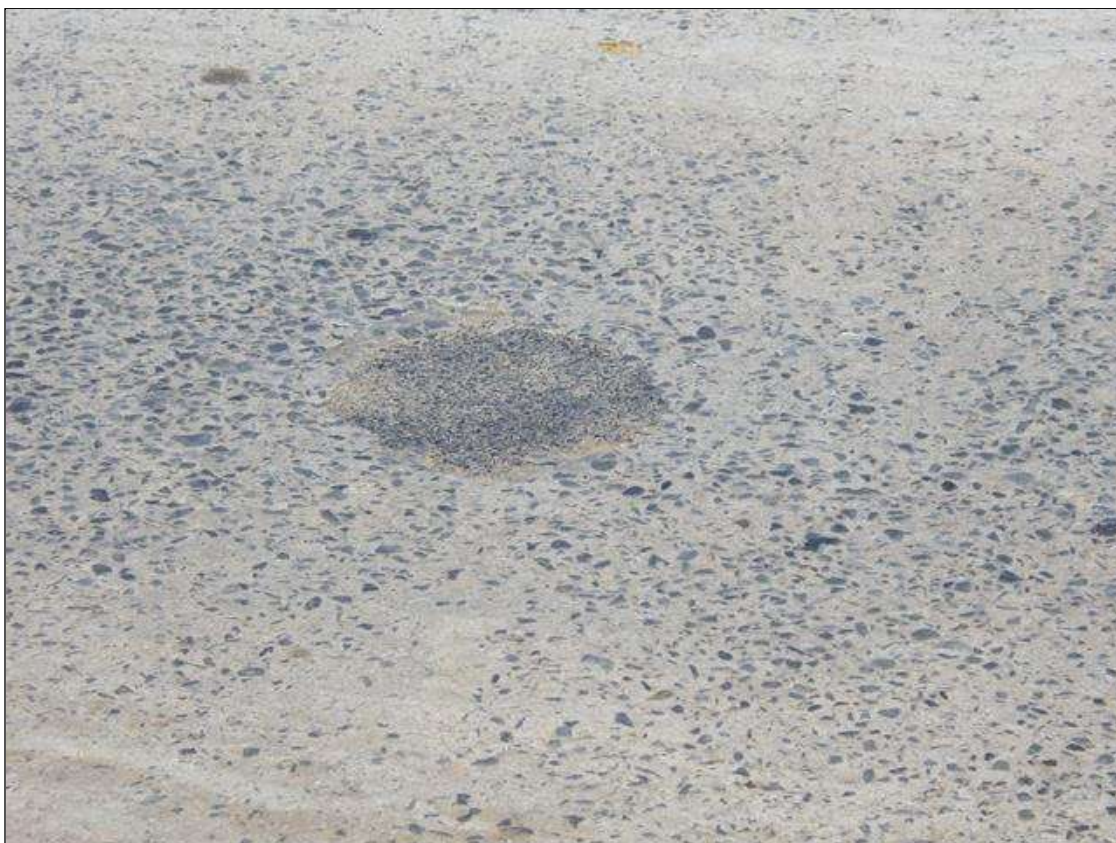
Span 3 Deck: 1 FOOT DIAMETER PATCHED AREA IN THE EASTBOUND LANE, 8 FEET FROM BENT 3
