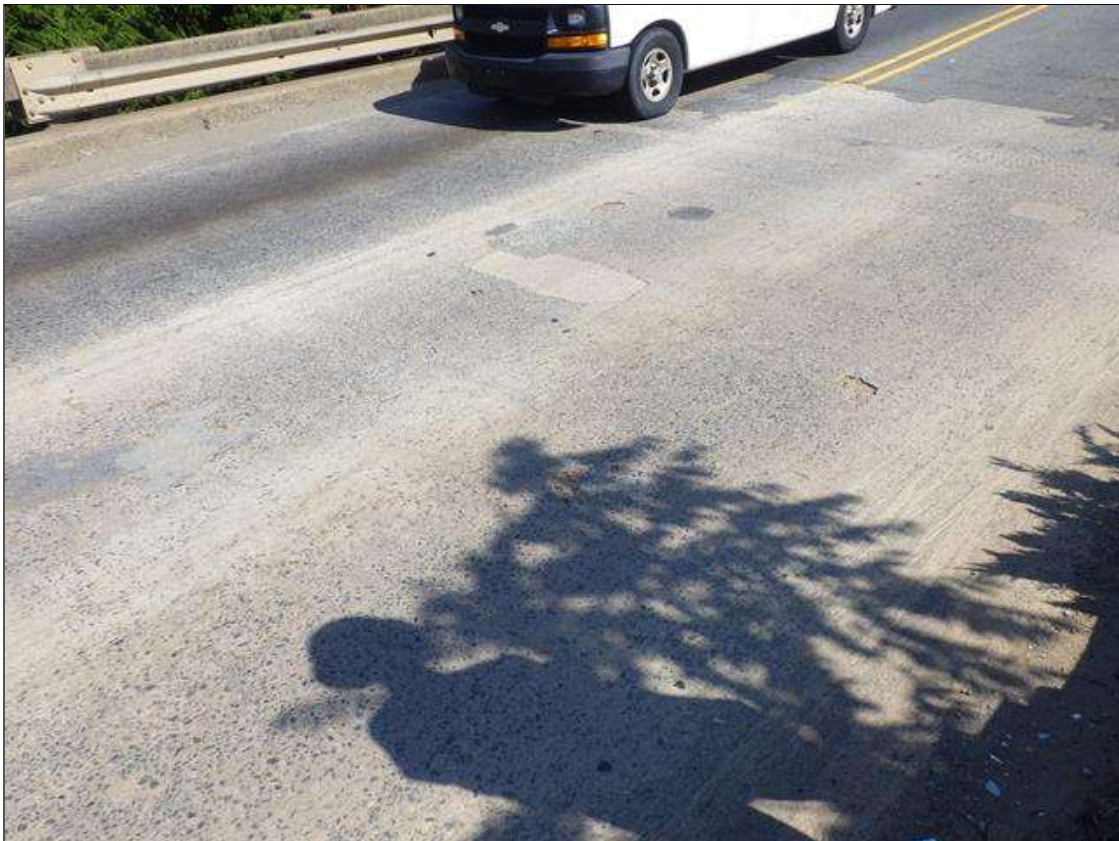
Span 4 Deck: (8) SPALLED AND DELAMINATED PATCHED AREAS UP TO 2 FEET 6 INCHES LONG X 2 FEET 6 INCHES WIDE X 1 INCH DEEP IN THE EASTBOUND LANE
