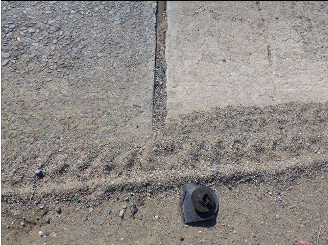
Span 4 Expansion Joint 3: FULL LENGTH LOOSE DEBRIS ACCUMULATION ALONG THE JOINT (OTHER JOINTS SIMILAR)
