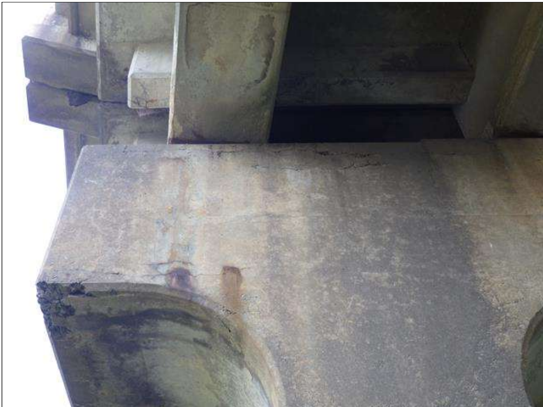
Bent 2 Cap 1: DELAMINATED AREA UP TO INTERMITTENT 7 FEET LONG X INTERMITTENT FULL HEIGHT X 1 FOOT WIDE WITH RUST STAINING IN THE UNDERSIDE AND WEST FACES BELOW GIRDER 1
