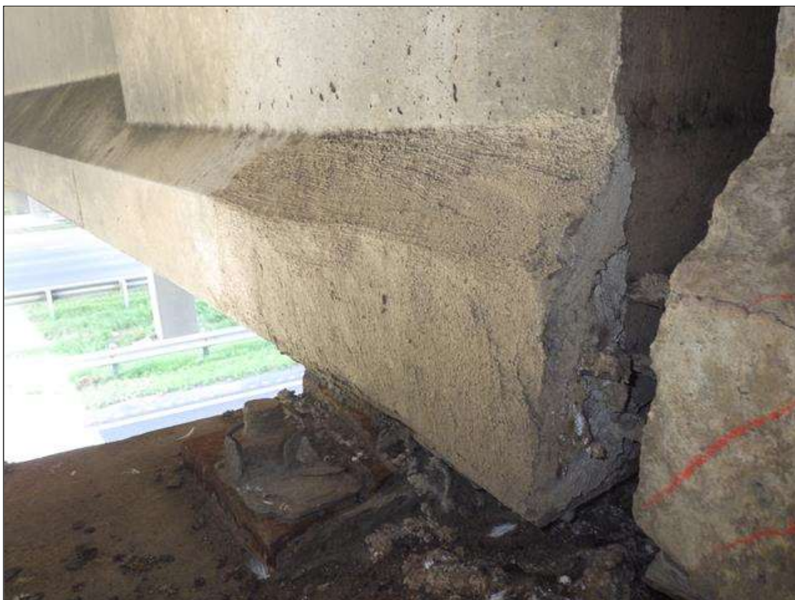
Span 3 Beam 3: PATCHED AREA UP TO 1 FOOT 8 INCHES LONG X 10 INCHES HIGH X 3 INCHES WIDE IN THE RIGHT BOTTOM FLANGE AT BENT 3
