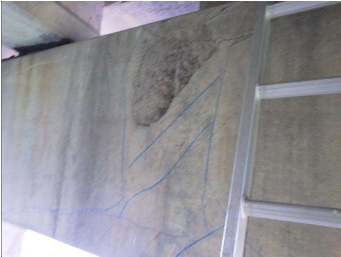
Bent 1 Cap 1: DELAMINATED AND SPALLED AREA UP TO 2 INCHES LONG X FULL HEIGHT X FULL WIDTH WITH EXPOSED REINFORCEMENT IN THE UNDERSIDE AND WEST FACES BELOW BAY 2
