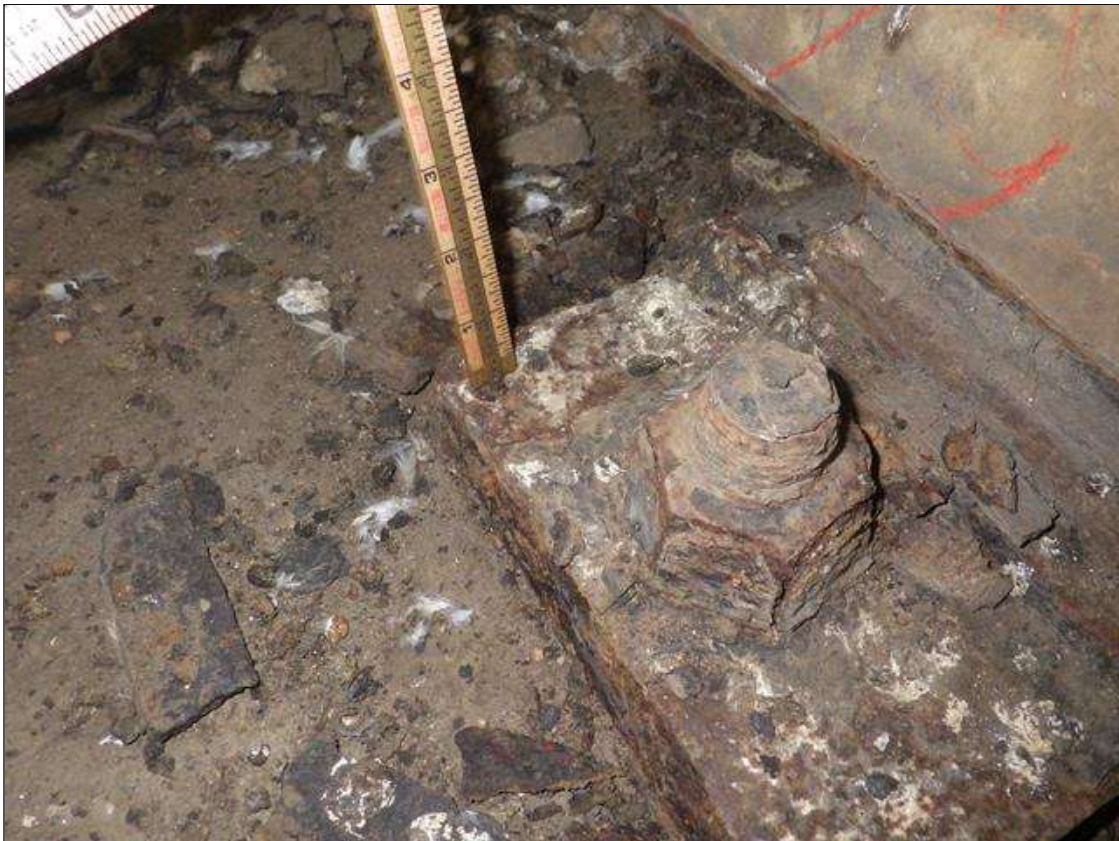
Span 4 Beam 3 - Near Bearing: ACTIVE CORROSION THROUGHOUT THE GIRDER 3 BEARING WITH 1/16 INCH SECTION LOSS (LESS THAN 25 PERCENT SECTION LOSS)
