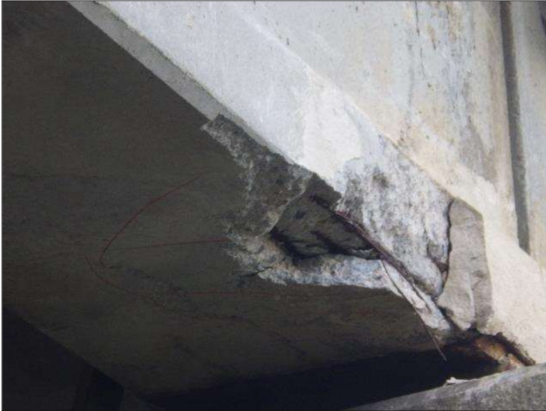
Span 4 Beam 1: 4 FEET LONG X 1 FOOT 2 INCHES WIDE X 7 INCHES HIGH X 2 INCHES DEEP SPALLED AND DELAMINATED PATCHED AREA IN THE LEFT BOTTOM FLANGE WITH (3) EXPOSED PRESTRESSING STRANDS, (1) STRAND SEVERED (PRIORITY ACTION REQUEST)
