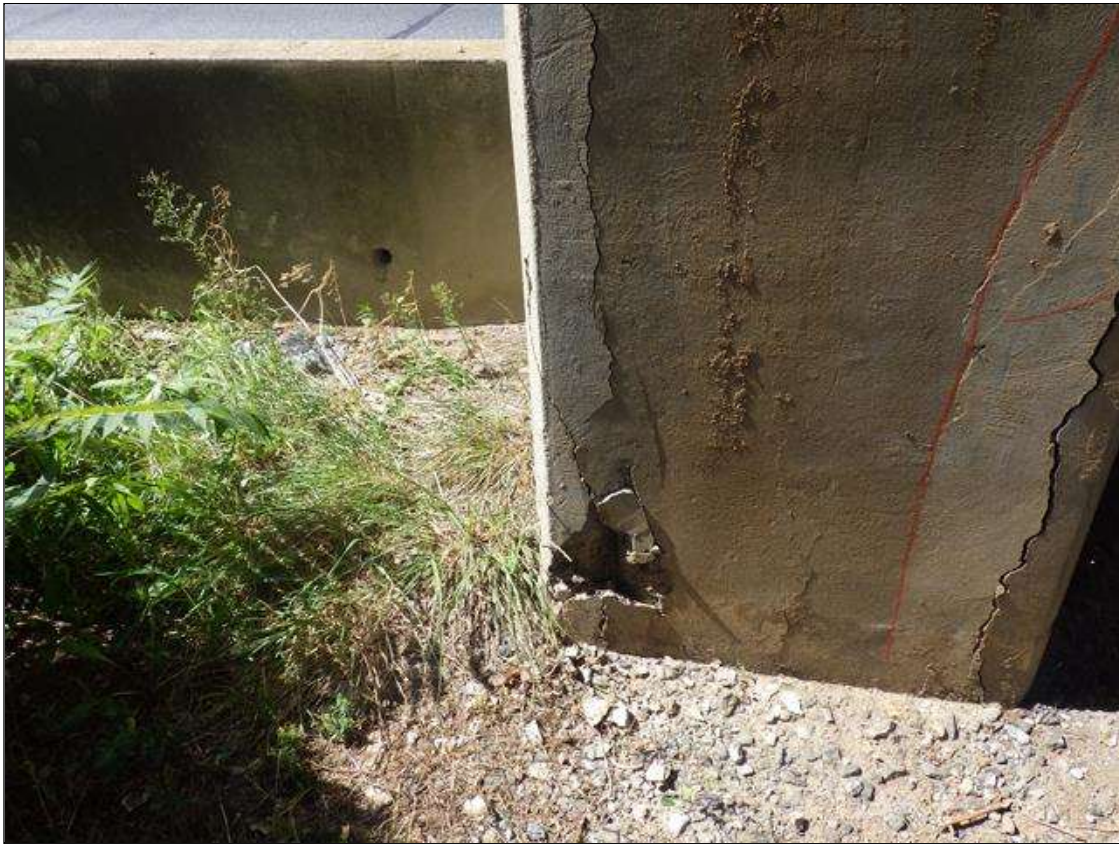
Bent 3 Pile 2: DELAMINATED AND SPALLED AREA UP TO FULL HEIGHT X 11 INCHES LONG X 9 INCHES WIDE WITH EXPOSED REINFORCEMENT IN THE SOUTHEAST CORNER
