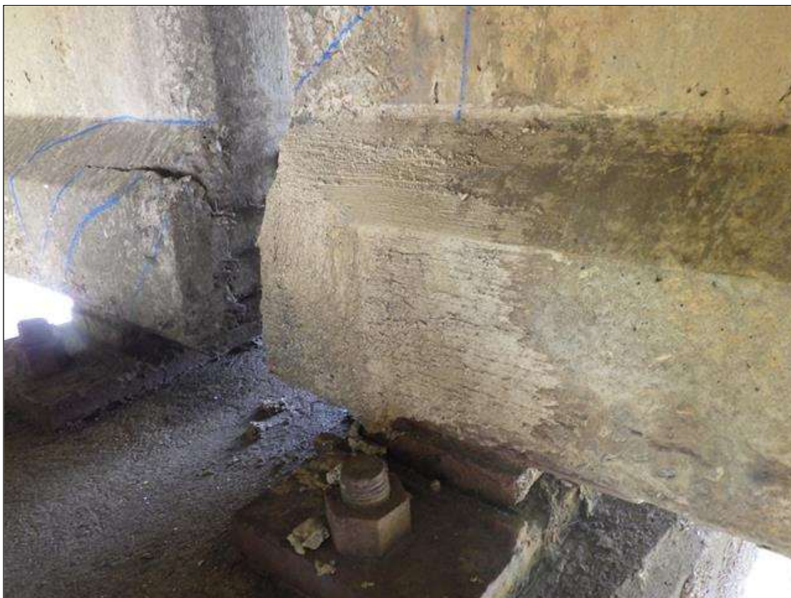
Span 2 Beam 3: PATCHED AREA UP TO 1 FOOT 3 INCHES LONG X 10 INCHES HIGH X 3 INCHES WIDE IN THE RIGHT BOTTOM FLANGE AT BENT 2
