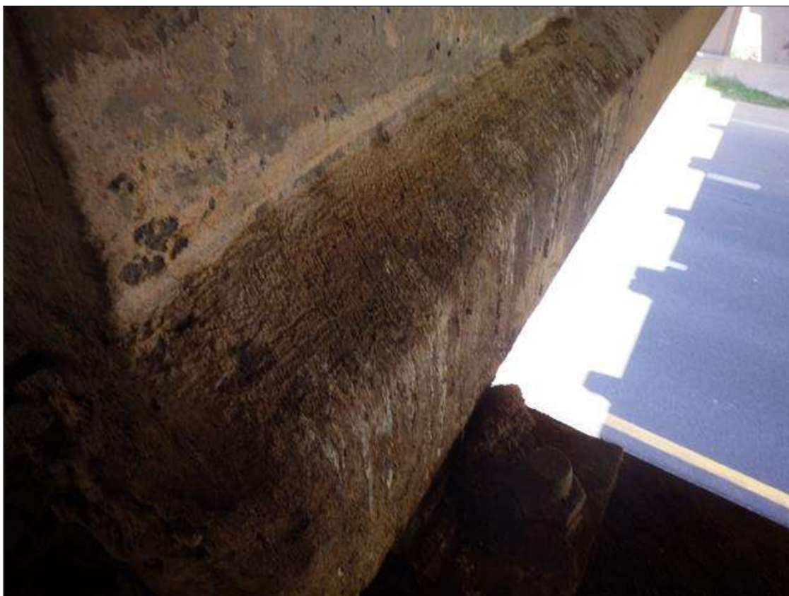
Span 2 Beam 4: PATCHED AREA UP TO 1 FOOT 4 INCHES LONG X 10 INCHES HIGH X 6 INCHES WIDE IN THE LEFT BOTTOM FLANGE AT BENT 2
