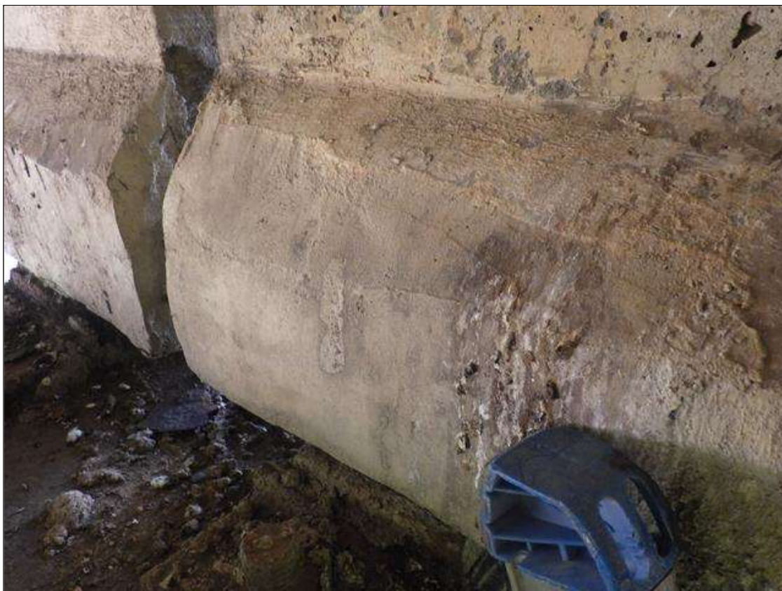
Span 4 Beam 1: PATCHED AREA UP TO 1 FOOT LONG X 9 INCHES HIGH X 3 INCHES WIDE IN THE RIGHT BOTTOM FLANGE AT BENT 3
