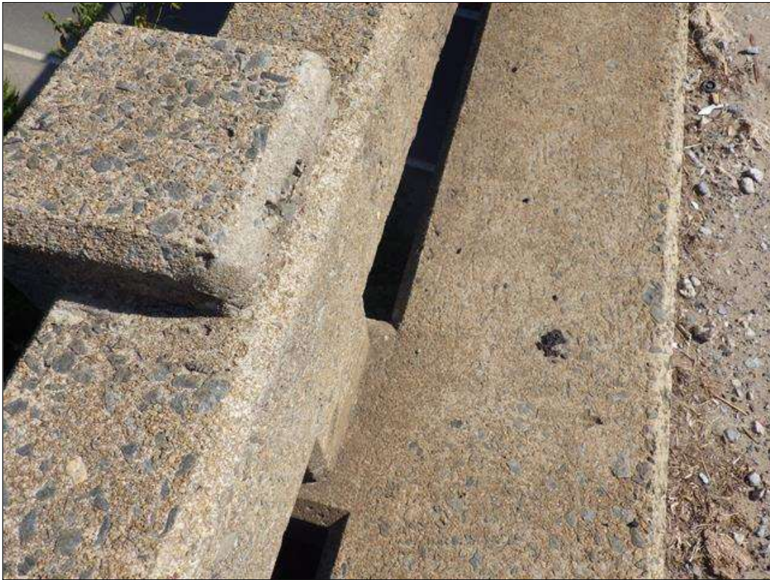
Span 1 Left Bridge Rail: EXPOSED SURFACE COARSE AGGREGATE THROUGHOUT THE RAIL AND CURB (OTHERS SIMILAR)
