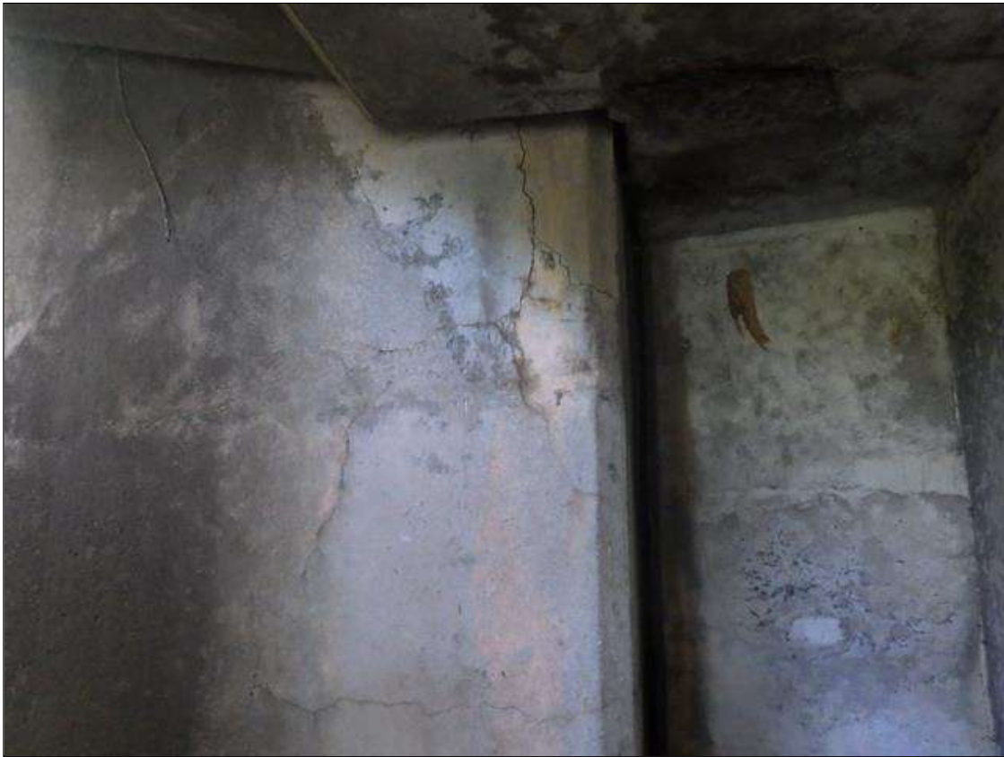
INTERMITTENT FULL HEIGHT X 5 INCHES LONG X 1 FOOT WIDE DELAMINATED AREA IN THE NORTHEAST WING WALL BELOW THE SOUTH OVERHANG
