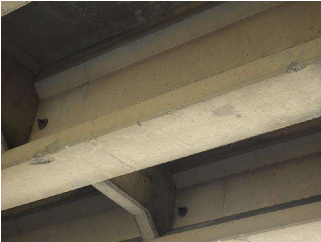
Span 2 Beam 3: (2) SPALLED AREAS UP TO 1 FOOT LONG X 4 INCHES WIDE X 4 INCHES HIGH IN THE LEFT BOTTOM FLANGE ABOVE THE MERGE ON RAMP LANE
