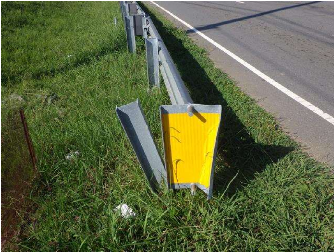
SOUTHEAST GUARDRAIL END TREATMENT
