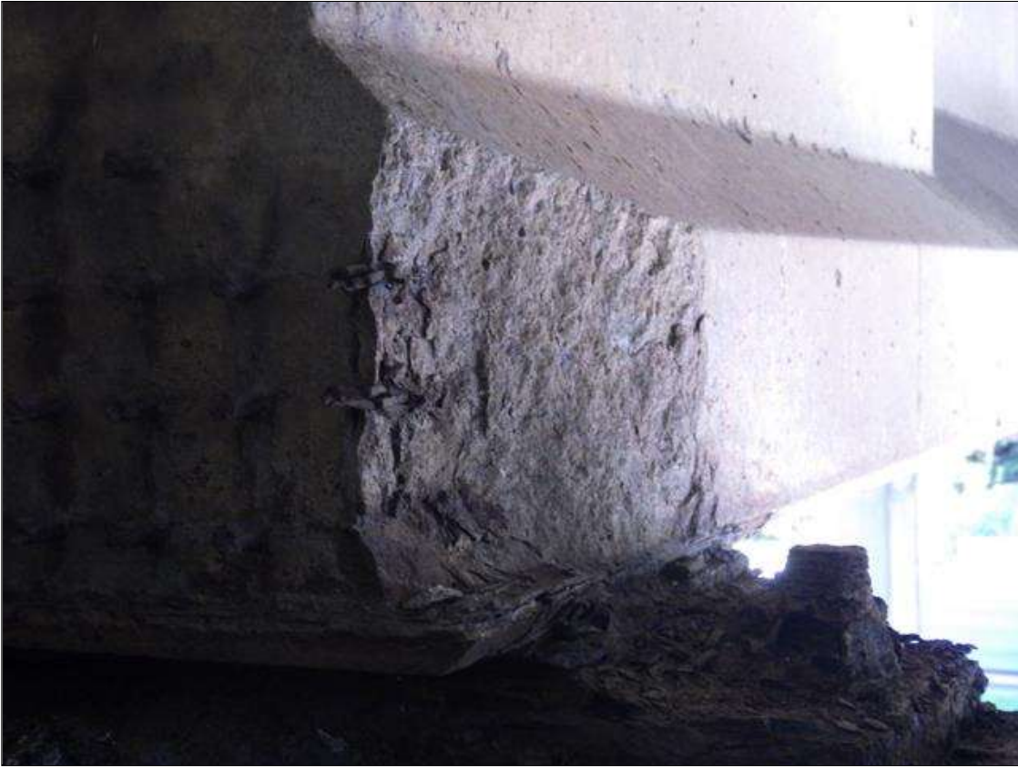
Span 2 Beam 4: 10 INCHES LONG X 10 INCHES HIGH X 2 INCHES WIDE SPALLED AREA WITH (3) EXPOSED PRESTRESSING STRANDS IN THE RIGHT BOTTOM FLANGE AT BENT 1 (PRIORITY ACTION REQUEST)
