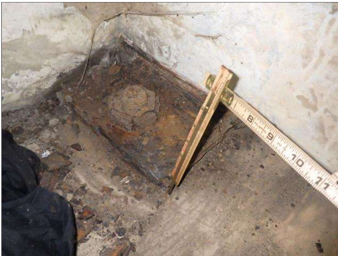
Span 4 Far Bearing: ACTIVE CORROSION THROUGHOUT THE GIRDER 4 BEARING WITH 1/16 INCH SECTION LOSS (LESS THAN 25 PERCENT SECTION LOSS)
