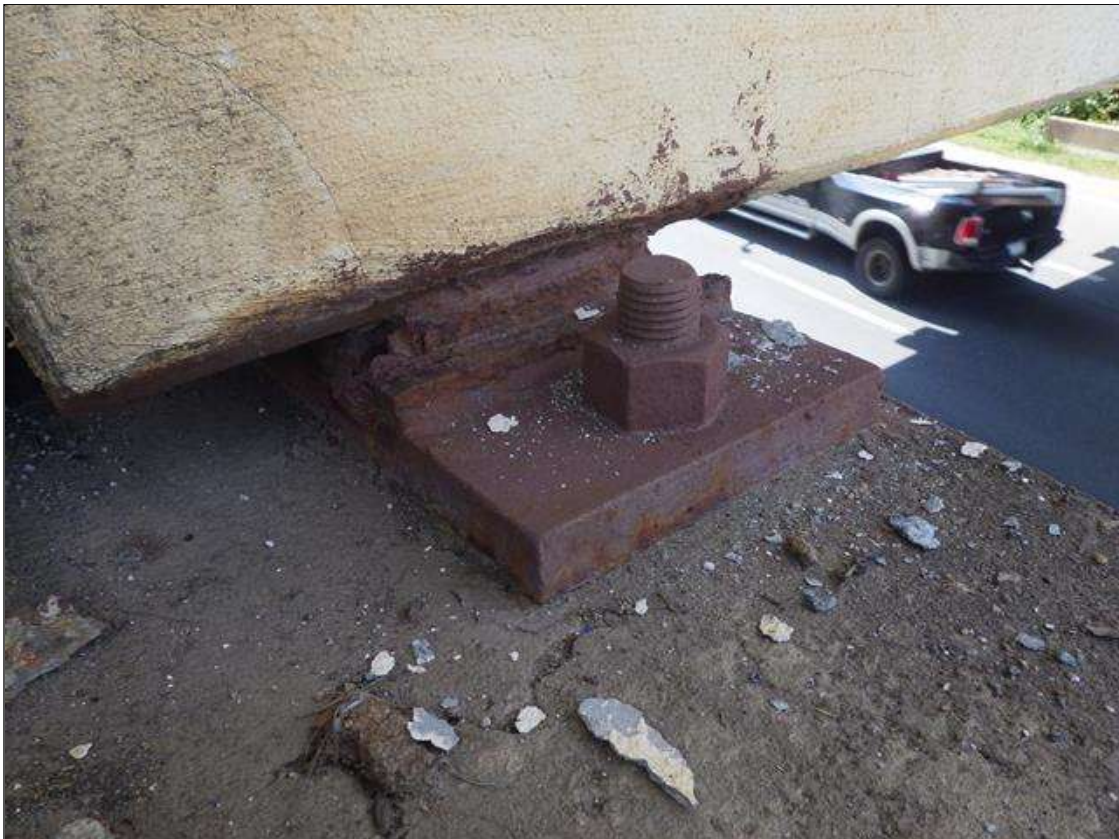
Span 2 Beam 1 - Far Bearing: ARRESTED SURFACE RUST UP TO FULL PERIMETER X FULL HEIGHT THROUGHOUT GIRDER 1 BEARING
