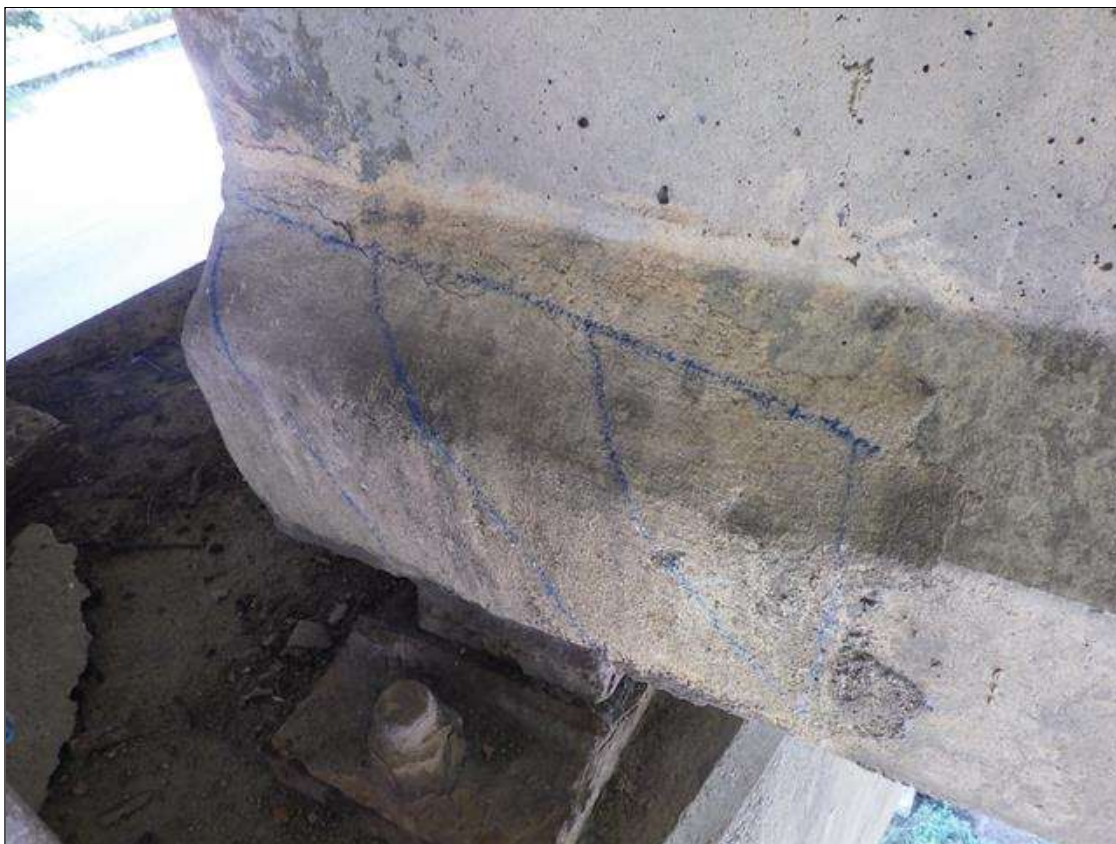
Span 3 Beam 3: DELAMINATED PATCH AREA UP TO 1 FOOT 3 INCHES LONG X 10 INCHES HIGH X 6 INCHES WIDE IN THE RIGHT BOTTOM FLANGE AT BENT 2
