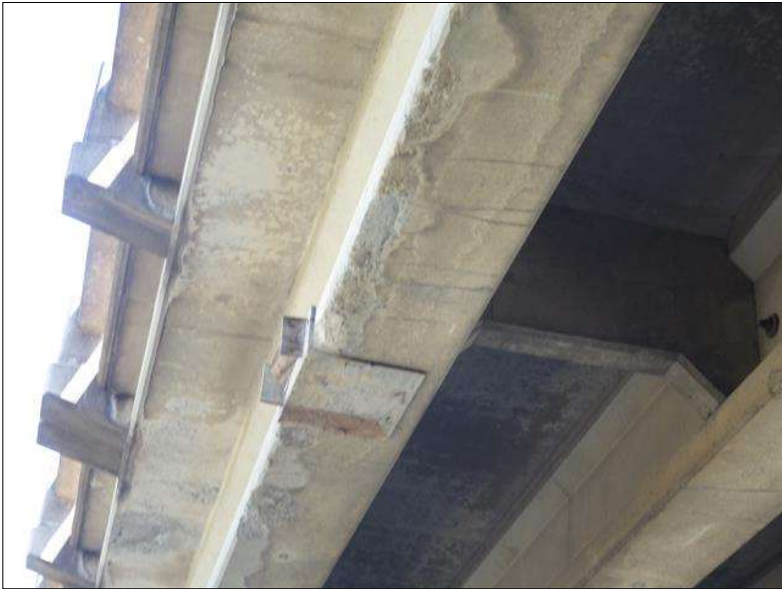
Span 2 Beam 1: SPALLED AREA UP TO INTERMITTENT 19 FEET LONG X 4 INCHES HIGH X 8 INCHES WIDE IN THE LEFT BOTTOM FLANGE, 12 FEET FROM BENT 1
