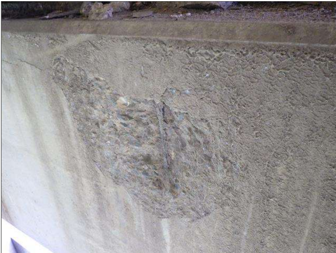
Bent 1 Cap 1: DELAMINATED AND SPALLED AREA UP TO 3 FEET LONG X 1 FOOT 4 INCHES HIGH X 1 INCH DEEP WITH EXPOSED REINFORCEMENT IN THE WEST FACE BELOW BAY 3
