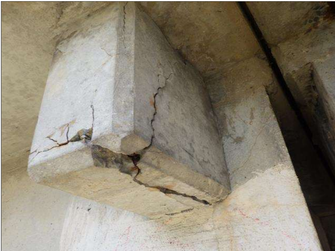
Span 2 Beam 5: DELAMINATED AND SPALLED AREA UP TO FULL LENGTH X FULL WIDTH X FULL HEIGHT WITH EXPOSED REINFORCEMENT IN THE END DIAPHRAGM BELOW THE SOUTH OVERHANG AT BENT 2
