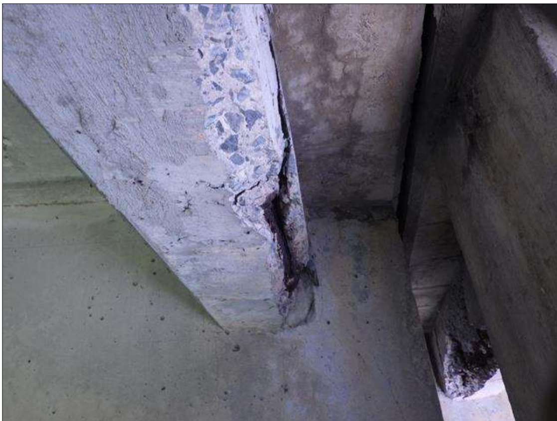
Span 1 Beam 3: DELAMINATED AND SPALLED AREA UP TO FULL LENGTH X FULL WIDTH X 4 INCHES HIGH WITH EXPOSED REINFORCEMENT IN BAY 3 END DIAPHRAGM AT BENT 1
