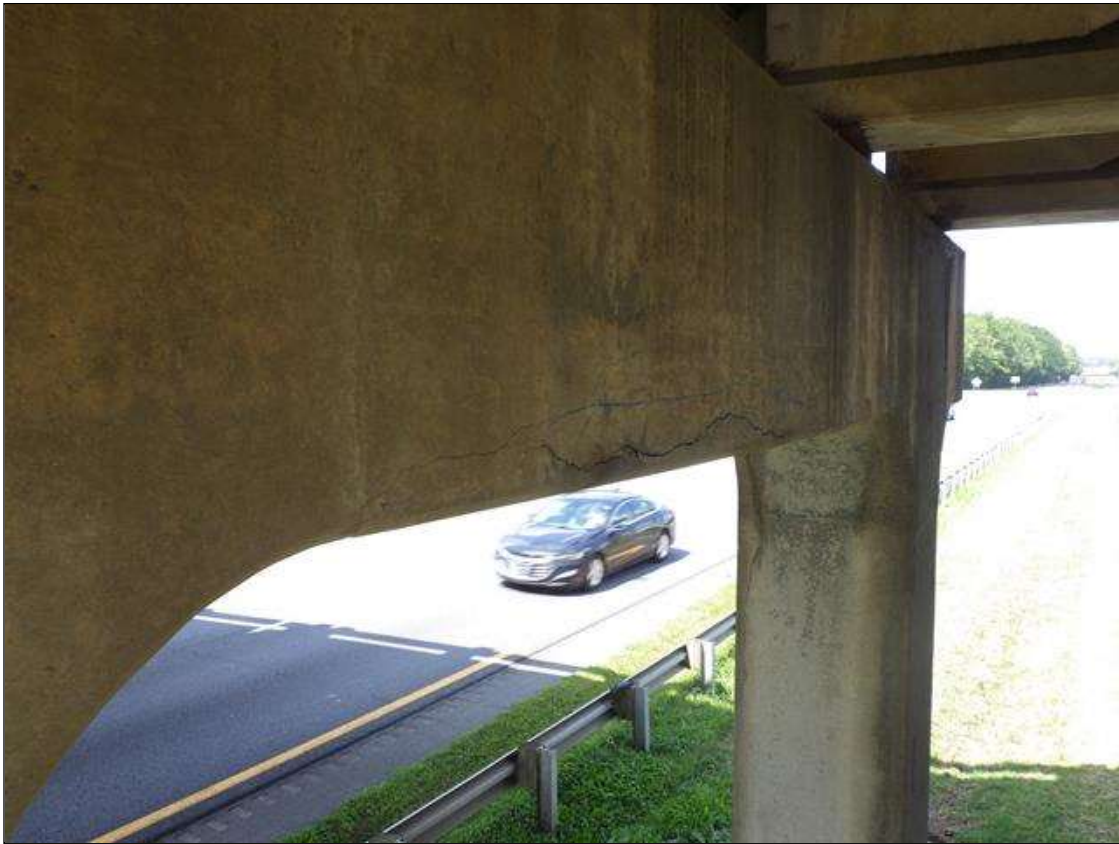
Bent 2 Cap 1: DELAMINATED AREA UP TO 13 FEET LONG X FULL WIDTH X 1 FOOT 6 INCHES HIGH WITH EFFLORESCENCE IN THE UNDERSIDE AND EAST FACES BETWEEN COLUMNS 1 AND 2
