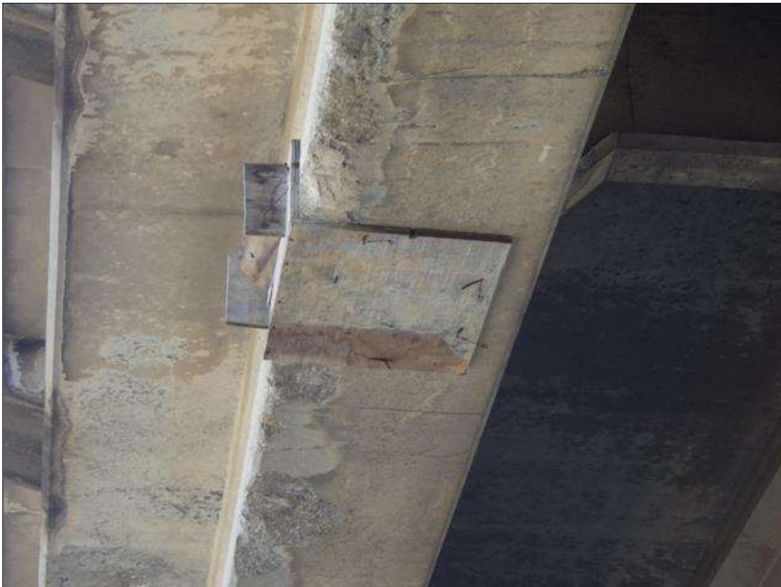
Span 2 Beam 2: (2) SPALLED AREAS UP TO 1 FOOT LONG X 4 INCHES WIDE X 3 INCHES HIGH IN THE LEFT BOTTOM FLANGE ABOVE THE MERGE ON RAMP LANE
