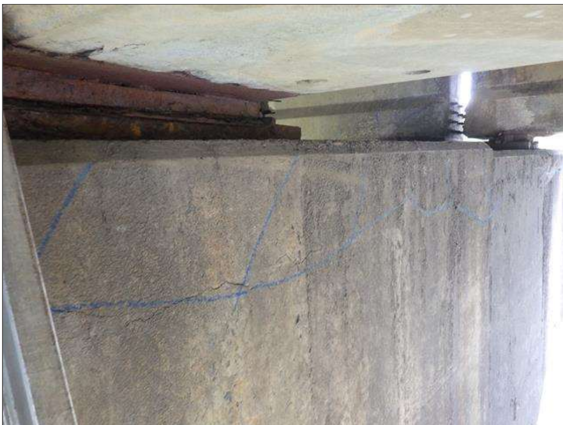
Bent 2 Cap 1: DELAMINATED AREA UP TO 11 FEET LONG X 1 FOOT HIGH X 3 INCHES WIDE IN THE EAST FACE BELOW BAY 2
