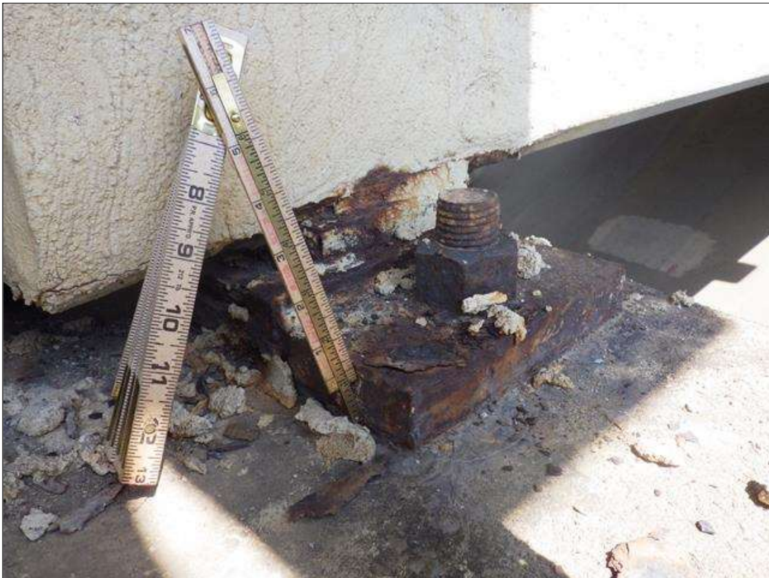
Span 4 Beam 4 - Near Bearing: ACTIVE CORROSION THROUGHOUT THE GIRDER 4 BEARING WITH 1/32 INCH SECTION LOSS
