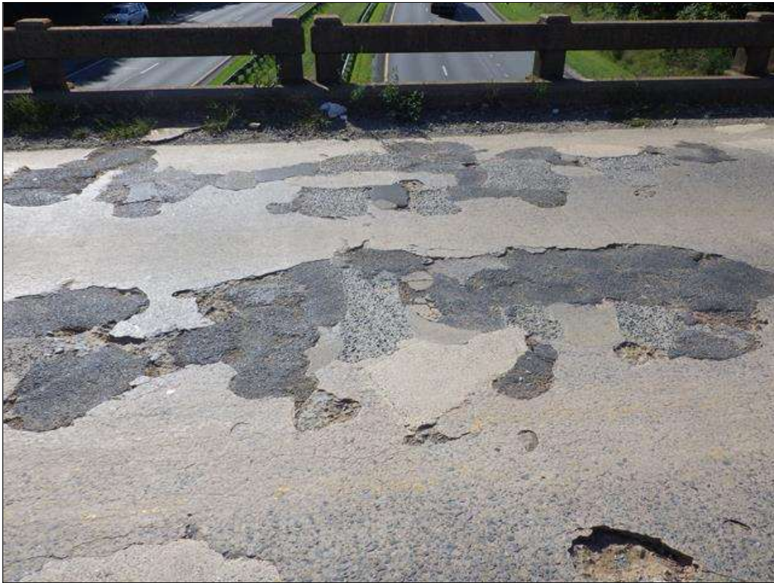
Span 2 Deck: INTERMITTENT FULL LENGTH X INTERMITTENT FULL WIDTH X UP TO 1 1/2 INCHES DEEP DELAMINATIONS, SPALLS, AND FAILED PATCHES THROUGHOUT THE DECK WITH 30 PERCENT OF DECK AREA AFFECTED
