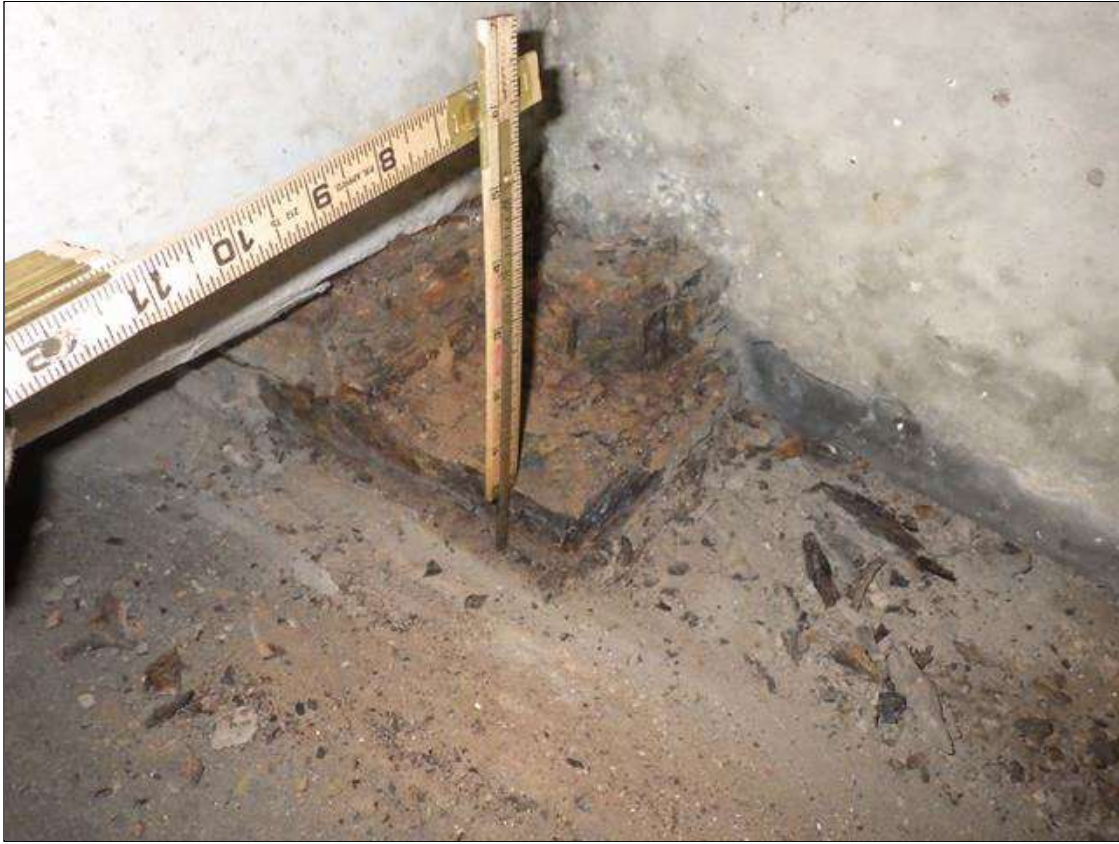
Span 1 Beam 4 - Near Bearing: ACTIVE CORROSION UP TO FULL PERIMETER X FULL HEIGHT WITH 1 1/4 INCHES REMAINING (GREATER THAN OR EQUAL TO 1/16 INCH SECTION LOSS AND LESS THAN 25 PERCENT SECTION LOSS) THROUGHOUT GIRDER 4 BEARING
