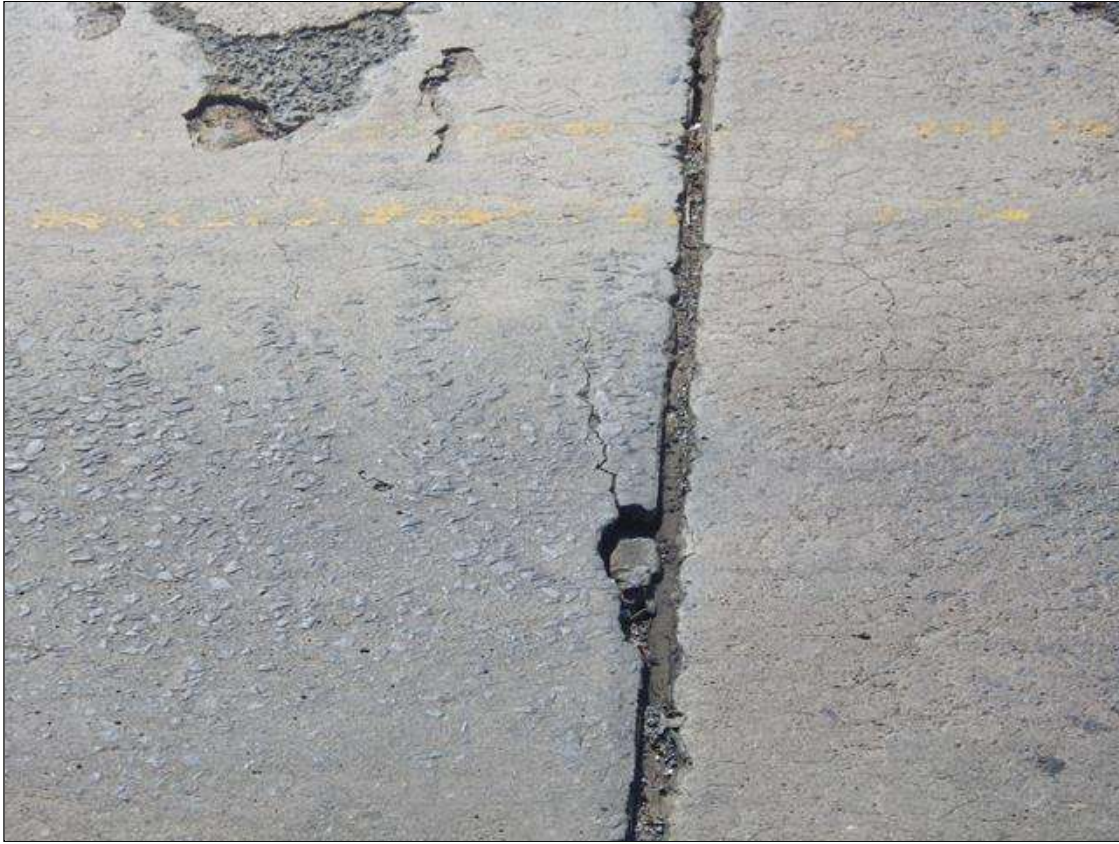
Span 3 Deck: 2 FEET 9 INCHES WIDE X 3 INCHES LONG X 1 1/2 INCHES DEEP SPALLED AND DELAMINATED AREA IN THE WESTBOUND LANE AT BENT 2
