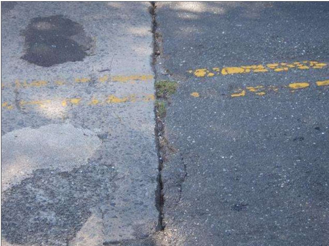
5 INCHES LONG X 15 FEET WIDE X 2 INCHES DEEP SPALLED AND DELAMINATED AREA IN THE WEST APPROACH ASPHALT WEARING SURFACE AT END BENT 1
