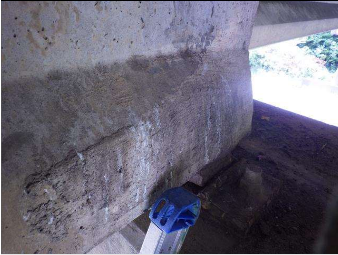
Span 3 Beam 3: PATCHED AREA UP TO 2 FEET LONG X 10 INCHES HIGH X 3 INCHES WIDE IN THE LEFT BOTTOM FLANGE AT BENT 2
