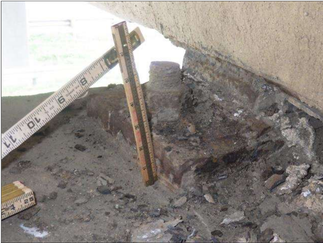
Span 3 Beam 3 - Far Bearing: ACTIVE CORROSION THROUGHOUT THE GIRDER 3 BEARING WITH 1/16 INCH SECTION LOSS (LESS THAN 25 PERCENT SECTION LOSS)
