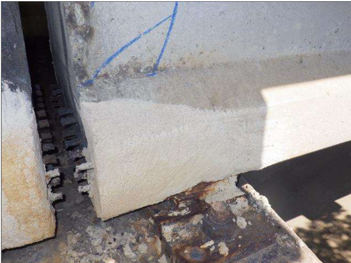
Span 4 Beam 4: PATCHED AREA UP TO 1 FOOT LONG X 10 INCHES HIGH X 3 INCHES WIDE IN THE BOTTOM RIGHT FLANGE AT BENT 3
