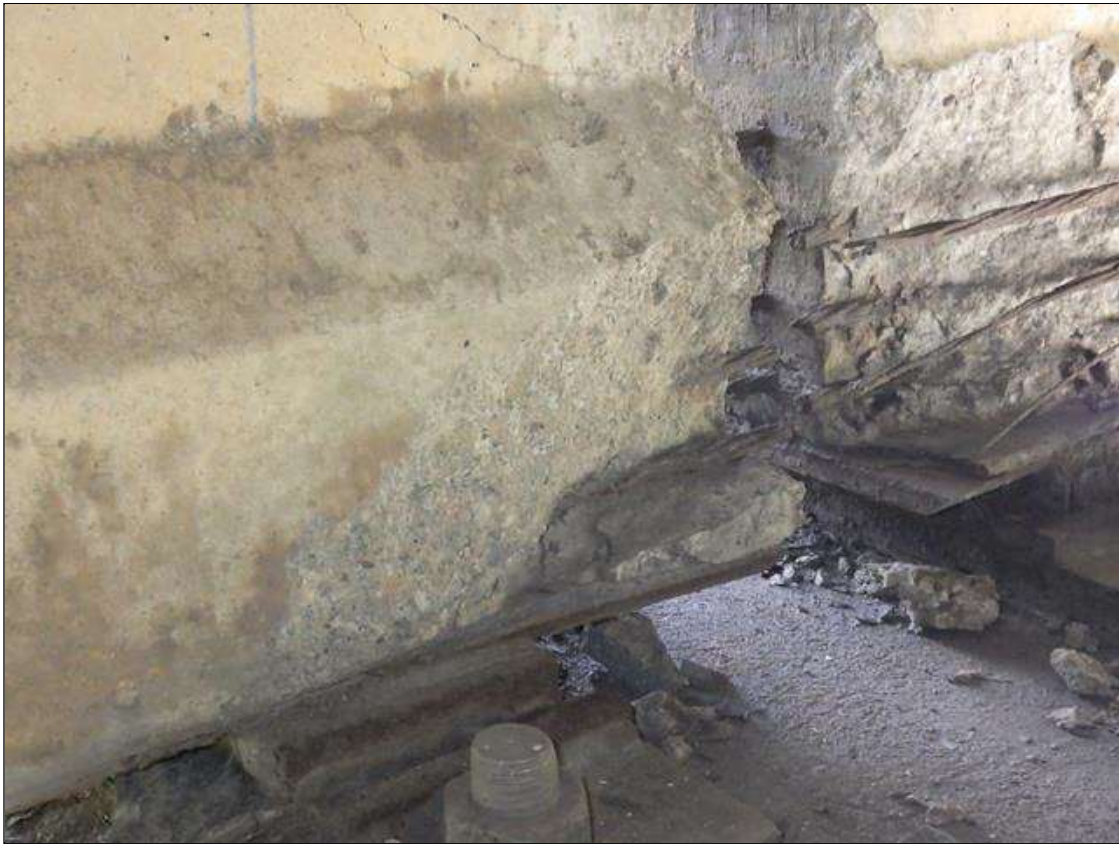
Span 1 Beam 1: 1 FOOT LONG X 8 INCHES HIGH X 3 INCHES WIDE SPALLED AREA WITH (2) EXPOSED PRESTRESSING STRANDS IN THE RIGHT BOTTOM FLANGE AT BENT 1 (PRIORITY ACTION REQUEST)
