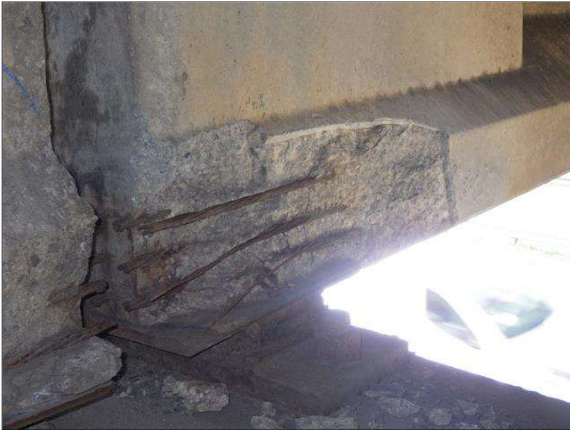
Span 2 Beam 1: 2 FEET 3 INCHES LONG X 10 INCHES HIGH X 4 INCHES WIDE SPALLED AREA WITH (6) EXPOSED PRESTRESSING STRANDS IN THE RIGHT BOTTOM FLANGE AT BENT 1 (PRIORITY ACTION REQUEST)
