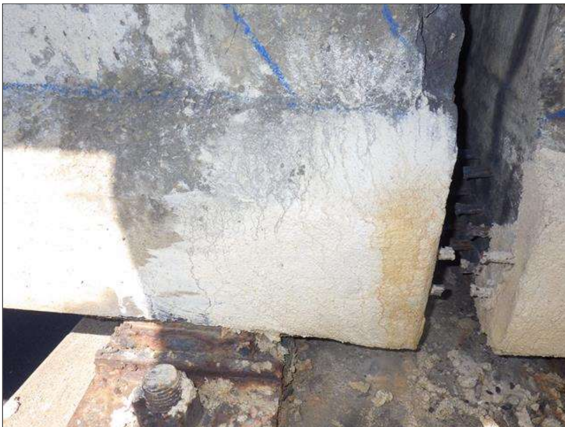
Span 3 Beam 4: PATCHED AREA UP TO 1 FOOT LONG X 10 INCHES HIGH X 3 INCHES WIDE IN THE BOTTOM RIGHT FLANGE AT BENT 3
