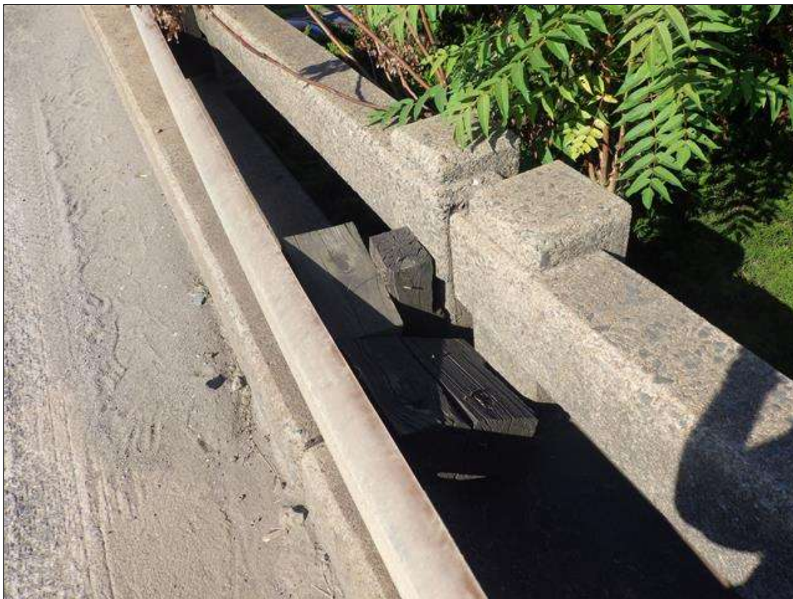
IMPACT DAMAGE TO THE NORTHEAST GUARDRAIL SPACER BLOCKS, 8 FEET FROM END BENT 2
