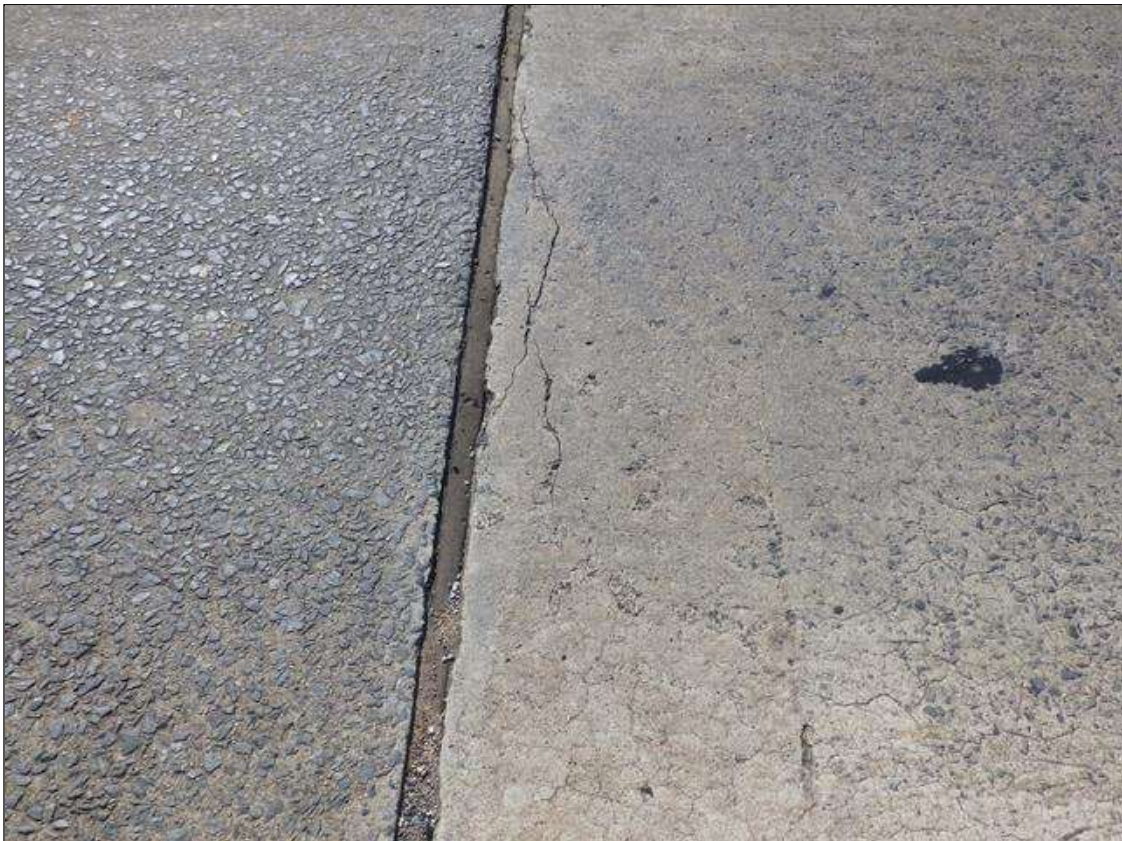
Span 3 Deck: INTERMITTENT 9 FEET WIDE X 6 INCHES LONG DELAMINATED AREA IN THE WESTBOUND LANE AT BENT 3
