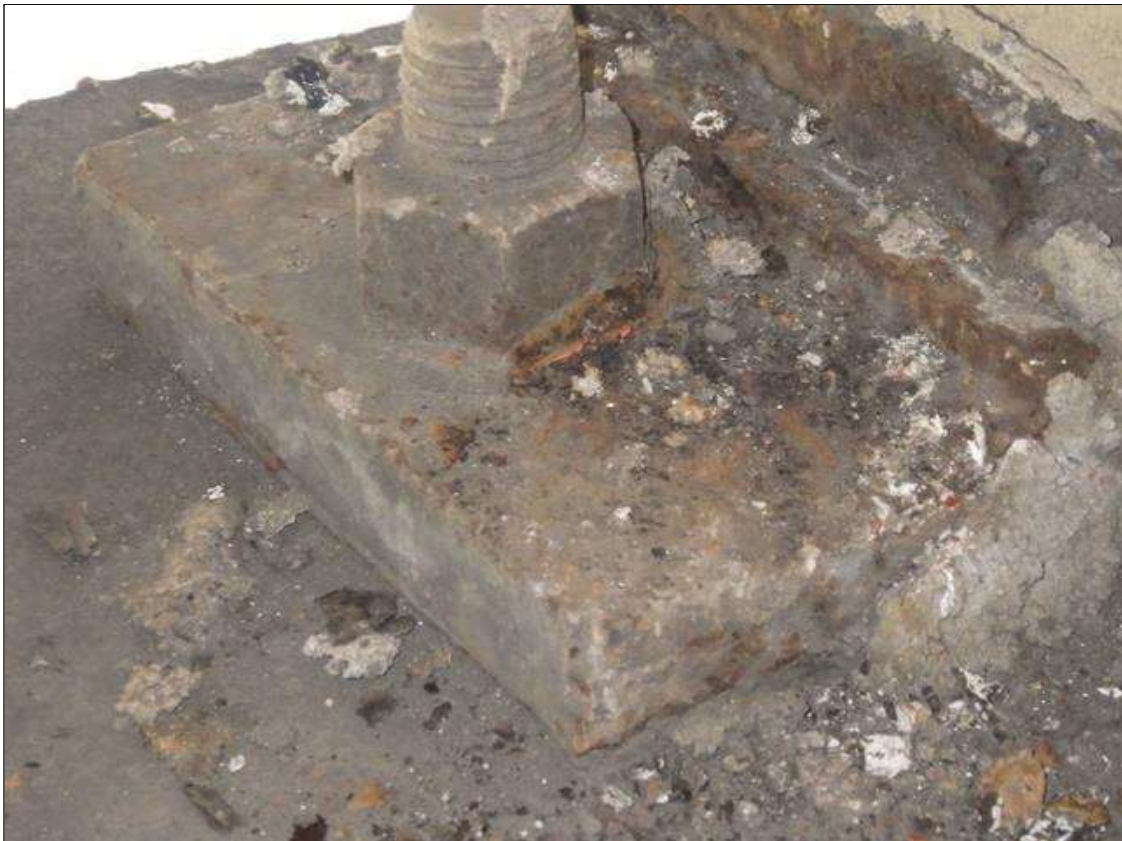
Span 3 Beam 1 - Far Bearing: SURFACE RUST THROUGHOUT THE GIRDER 1 BEARING
