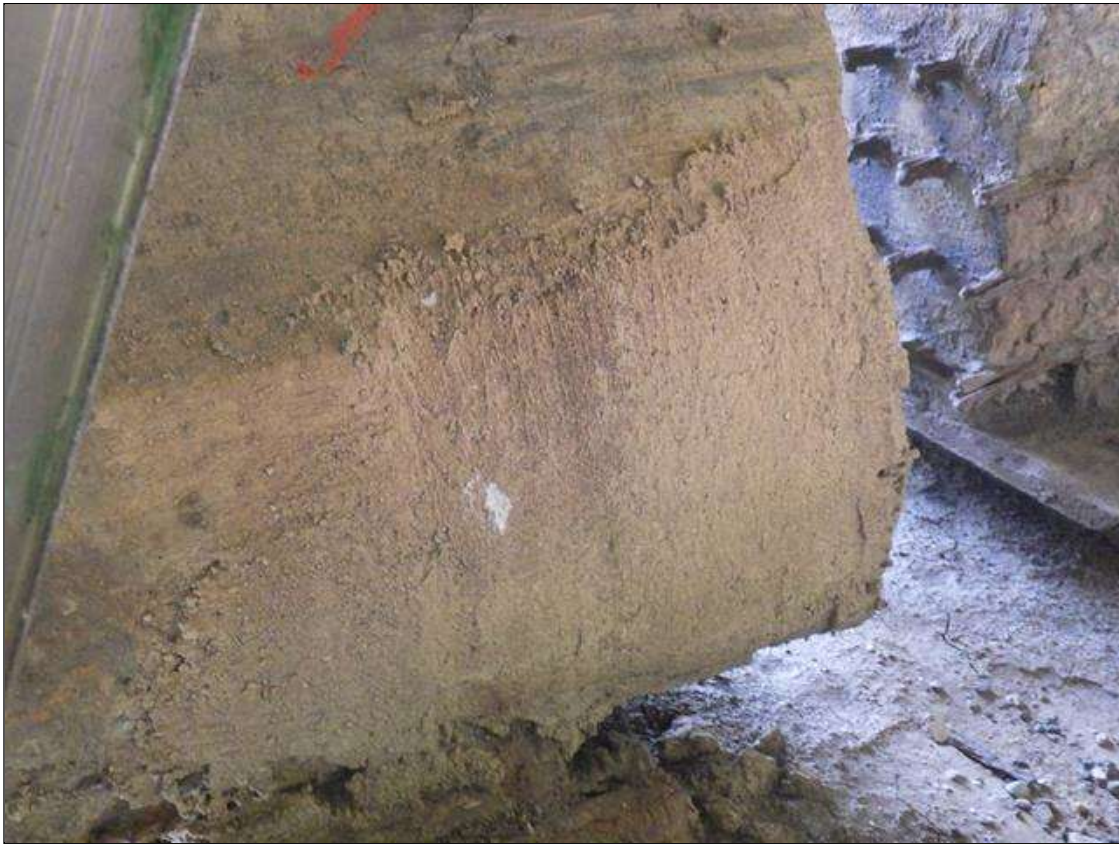
Span 3 Beam 4: PATCHED AREA UP TO 1 FOOT LONG X 10 INCHES HIGH X 3 INCHES WIDE IN THE LEFT BOTTOM FLANGE AT BENT 2
