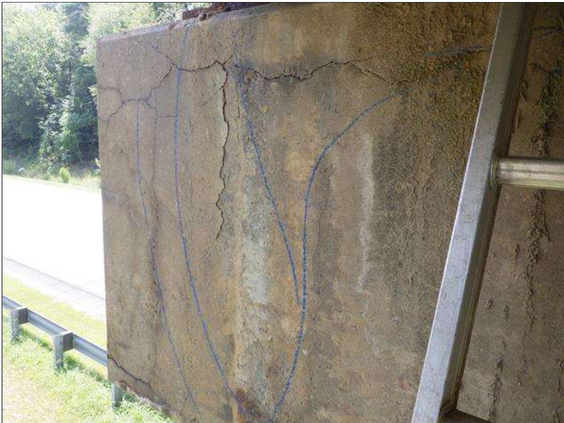
Bent 2 Cap 1: DELAMINATED AREA UP TO 6 FEET 6 INCHES LONG X FULL WIDTH X FULL HEIGHT WITH EFFLORESCENCE IN THE SOUTH AND EAST FACES BELOW GIRDER 4
