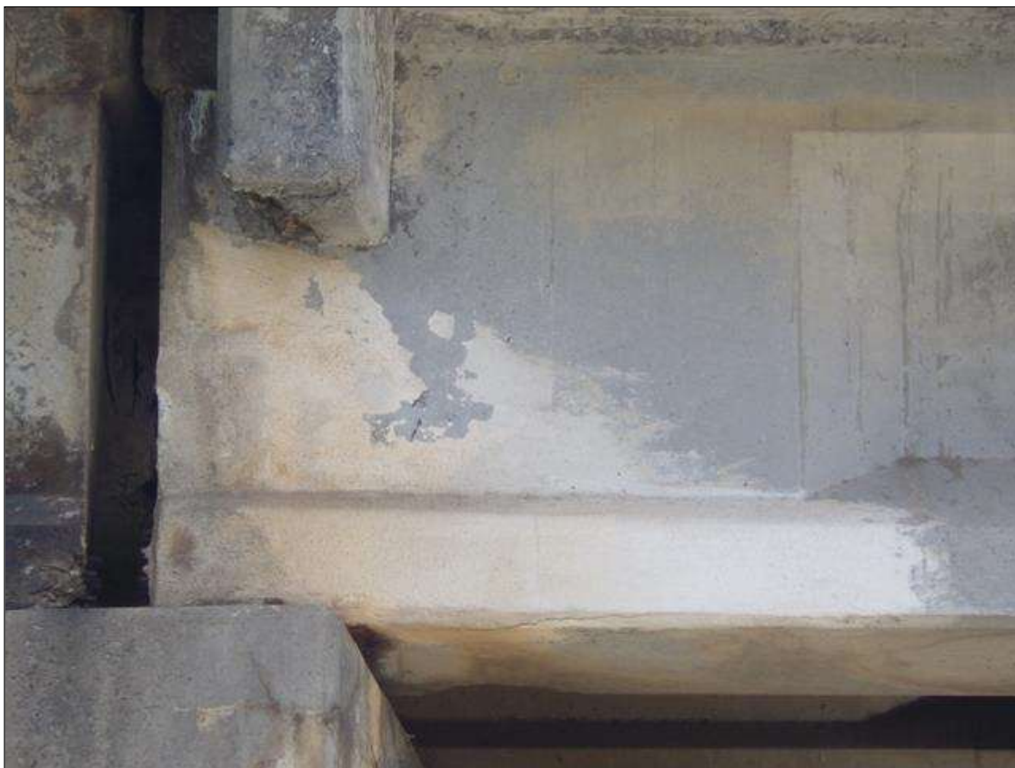
Span 2 Beam 2: PATCHED AREA UP TO 4 FEET LONG X 2 FEET 10 INCHES LONG X 3 INCHES WIDE IN THE RIGHT FACE OF THE WEB AND BOTTOM FLANGE AT BENT 1
