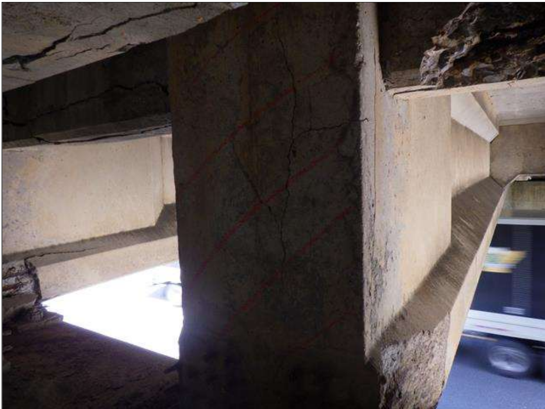
Span 2 Beam 3: DELAMINATED AREA UP TO 2 INCHES LONG X FULL HEIGHT X FULL WIDTH IN THE WEST FACE OF THE WEB AND FLANGES AT BENT 1
