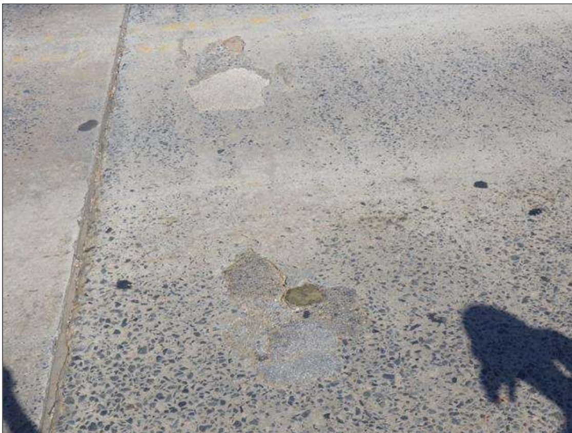
Span 3 Deck: 1 FOOT 4 INCHES LONG X 2 FEET 2 INCHES WIDE X 1 INCH DEEP SPALLED AND DELAMINATED PATCHED AREA IN THE EASTBOUND LANE, 2 FEET FROM BENT 2
