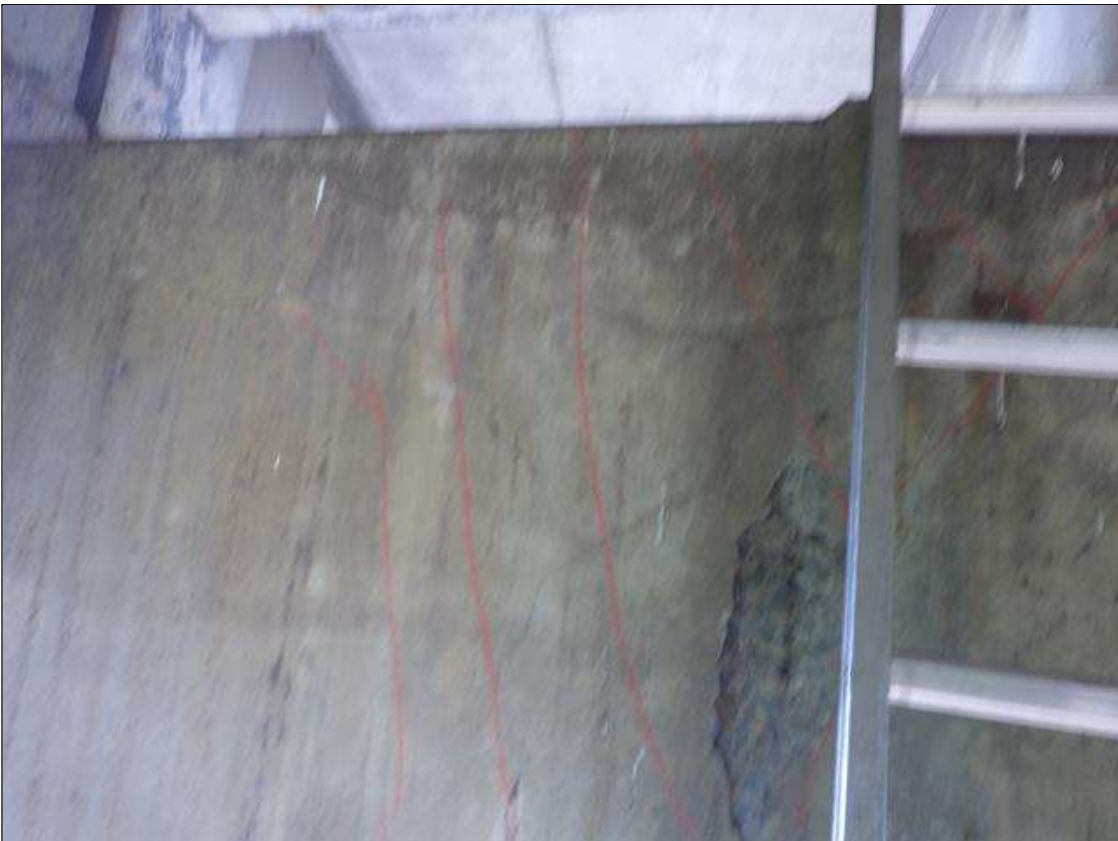
Bent 3 Cap 1: DELMINATED AND SPALLED AREA UP TO INTERMITTENT 9 FEET LONG X 3 FEET 1 INCH HIGH X 1 INCHES DEEP IN THE EAST FACE BELOW BAY 3 TO SOUTH OVERHANG
