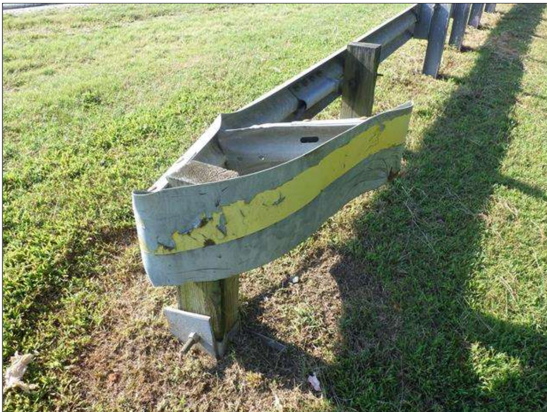
2 FEET LONG IMPACT DAMAGE TO THE NORTHEAST GUARDRAIL END TREATMENT
