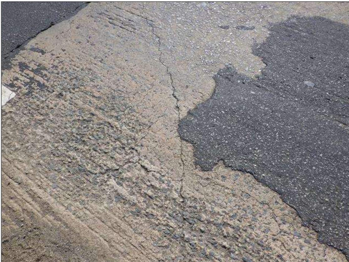
Span 4 Deck: 6 FEET 6 INCHES LONG X UP TO 1/8 INCH WIDE DIAGONAL CRACK IN THE WESTBOUND LANE AT END BENT 2
