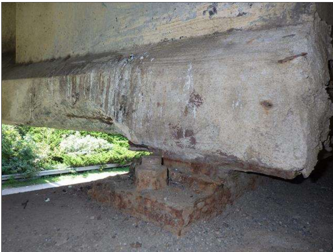
Span 2 Beam 3: 3 FOOT LONG X 10 INCHES HIGH X 10 INCHES WIDE SPALLED AREA WITH (1) EXPOSED PRESTRESSING STRAND IN THE RIGHT BOTTOM FLANGE AT BENT 2 (PRIORITY ACTION REQUEST)
