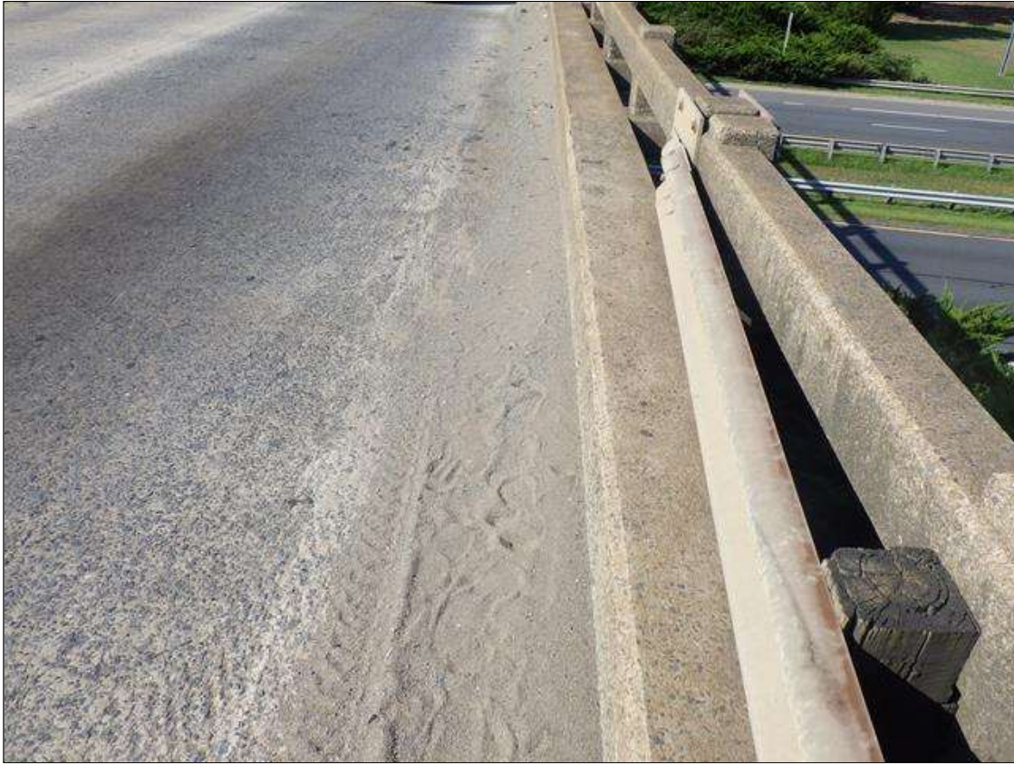
FULL LENGTH X UP TO 2 FEET WIDE DEBRIS BUILD-UP ALONG THE NORTH AND SOUTH BRIDGE RAILS
