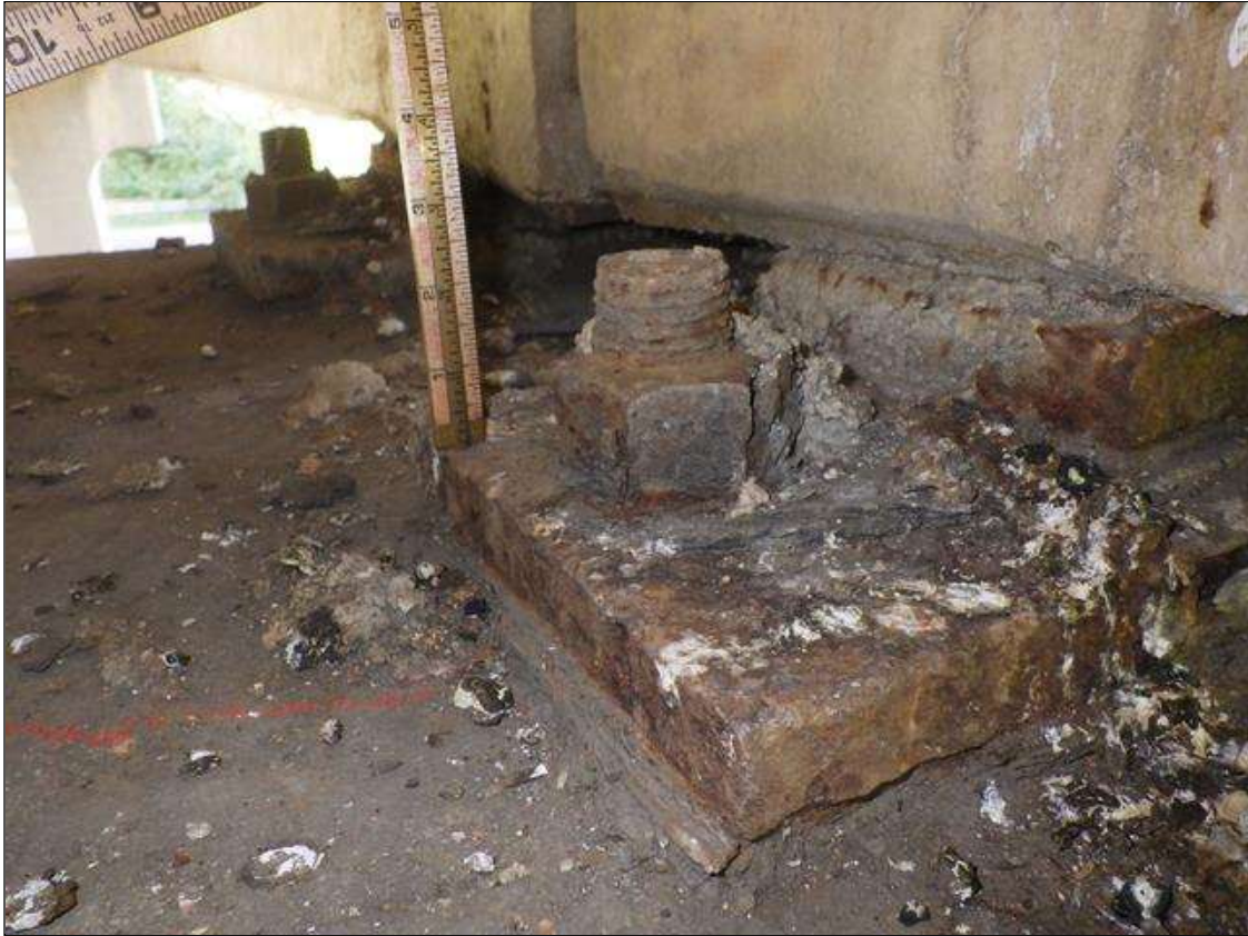
Span 4 Beam 1 - Near Bearing: ACTIVE CORROSION THROUGHOUT THE GIRDER 1 BEARING WITH 1/16 INCH SECTION LOSS (LESS THAN 25 PERCENT SECTION LOSS)
