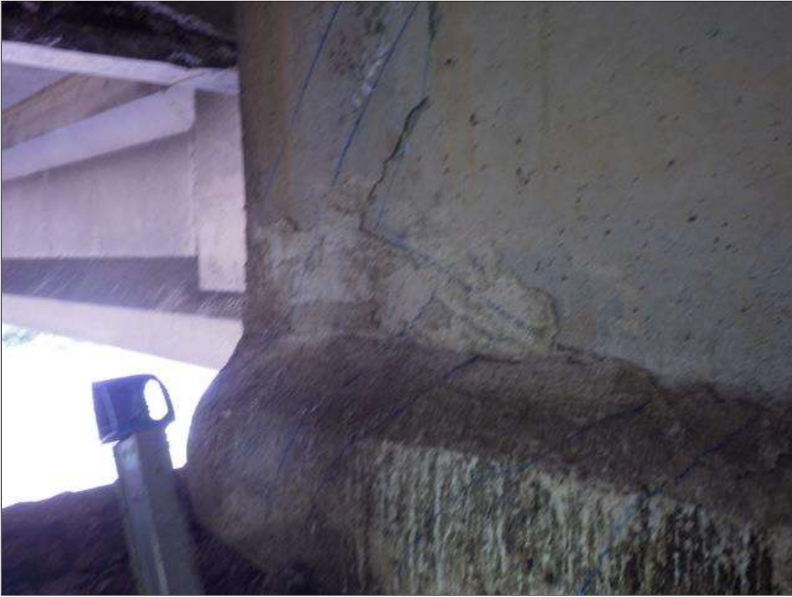
Span 1 Beam 3: DELAMINATED PATCH AREA UP TO 1 FOOT 9 INCHES LONG X FULL HEIGHT X 9 INCHES WIDE IN THE LEFT FACE OF THE WEB AND BOTTOM FLANGE AT BENT 1
