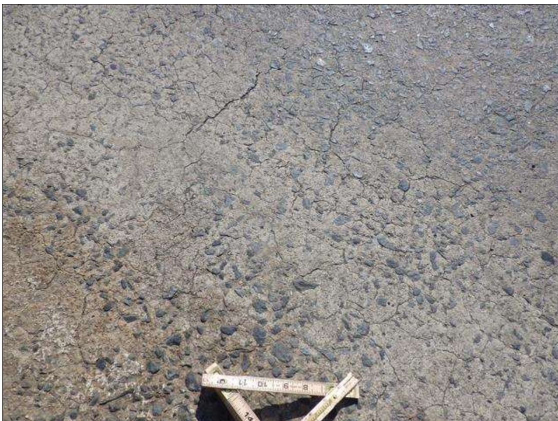
Span 1 Deck: FULL LENGTH X FULL WIDTH MAP CRACKING UP TO 1/8 INCH WIDE THROUGHOUT THE TOP OF THE DECK
