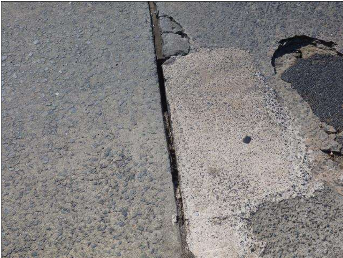
Span 3 Expansion Joint 2: 3 FEET LONG X FULL DEPTH MISSING JOINT MATERIAL IN THE WESTBOUND LANE
