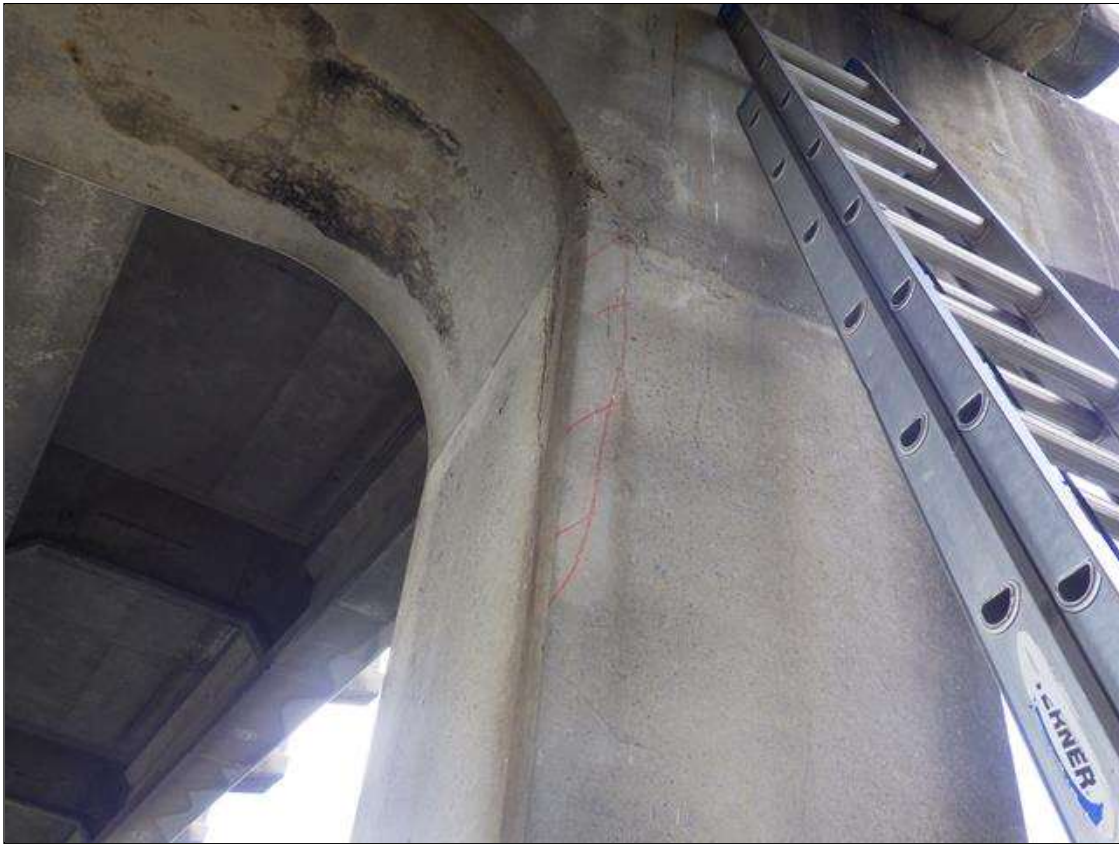
Bent 3 Pile 1: DELAMINATED AREA UP TO 3 FEET 4 INCHES HIGH X 4 INCHES LONG X 5 INCHES WIDE IN THE SOUTHEAST CORNER ADJACENT TO BOTTOM OF CAP
