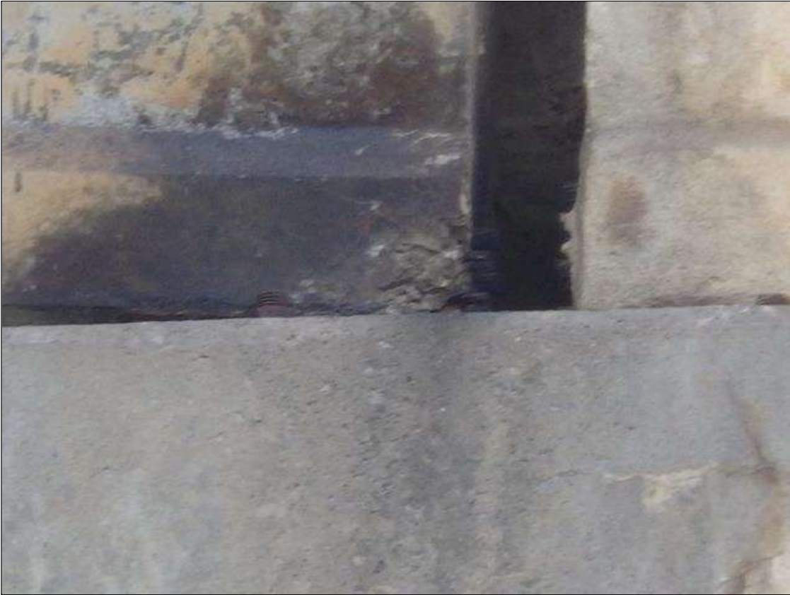
Span 1 Beam 4: 9 INCHES LONG X 5 INCHES HIGH X 3 INCHES WIDE SPALLED AREA WITH (1) EXPOSED PRESTRESSING STRAND IN THE RIGHT BOTTOM FLANGE AT BENT 1 (PRIORITY ACTION REQUEST)
