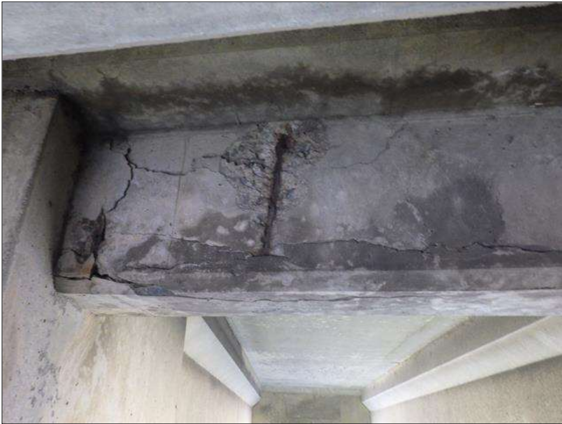
Span 2 Beam 2: DELAMINATED AND SPALLED AREA UP TO FULL LENGTH X FULL WIDTH X FULL HEIGHT WITH EXPOSED REINFORCEMENT IN BAY 2 END DIAPHRAGM AT BENT 2
