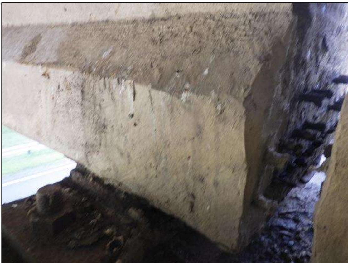
Span 3 Beam 1: PATCHED AREA UP TO 1 FOOT LONG X 9 INCHES HIGH X 3 INCHES WIDE IN THE RIGHT BOTTOM FLANGE AT BENT 3
