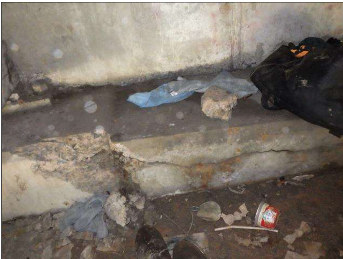
End Bent 2 Cap 1: 5 FEET 9 INCHES LONG X 1 FOOT HIGH X 1 FOOT WIDE SPALLED AND DELAMINATED AREA WITH EXPOSED REINFORCEMENT IN THE CAP BELOW BAY 3
