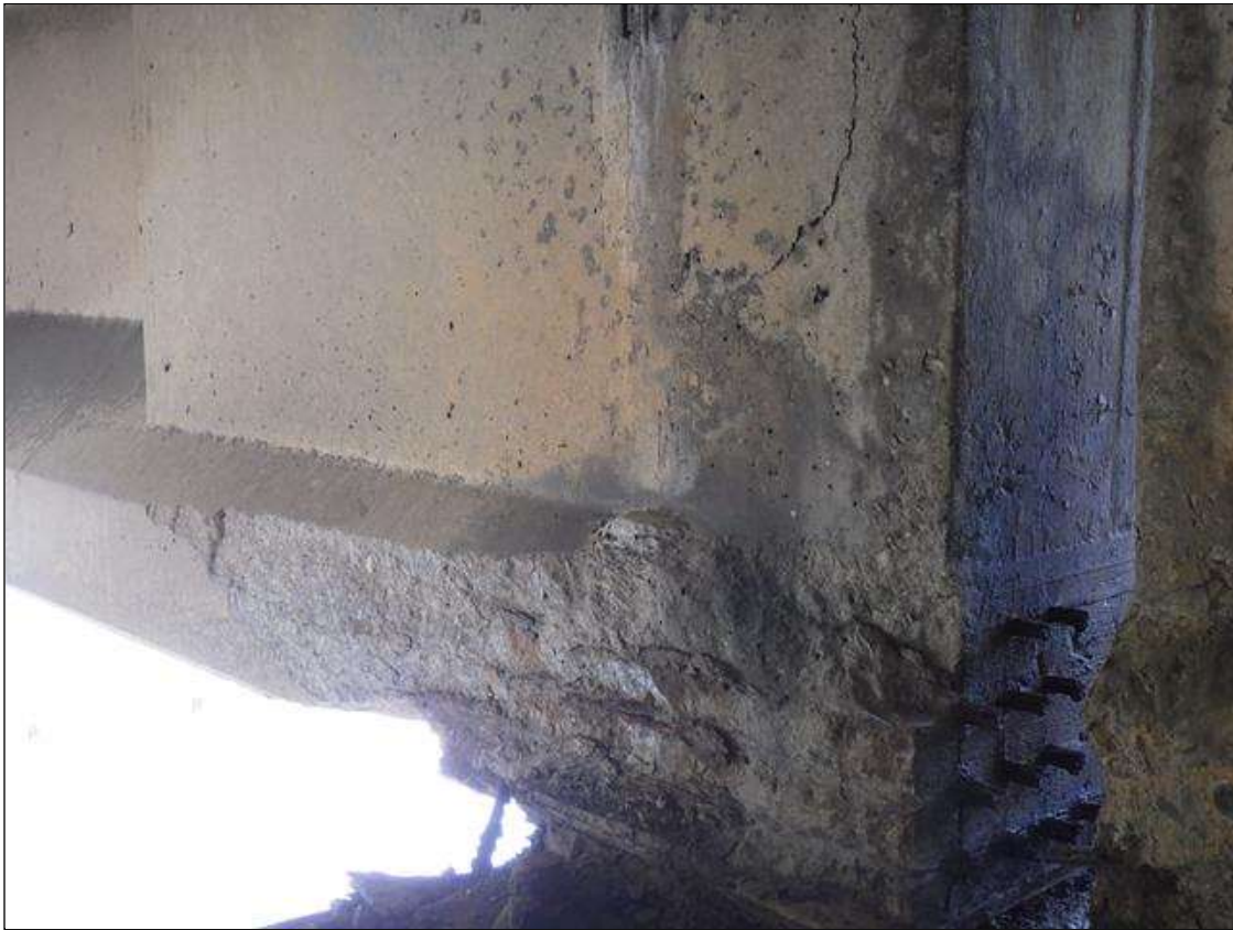
Span 2 Beam 5: 3 FEET 4 INCHES LONG X FULL HEIGHT X 4 INCHES WIDE SPALLED AND DELAMINATED AREA WITH (2) EXPOSED PRESTRESSING STRANDS IN THE LEFT BOTTOM FLANGE AND WEB AT BENT 1 (PRIORITY ACTION REQUEST)
