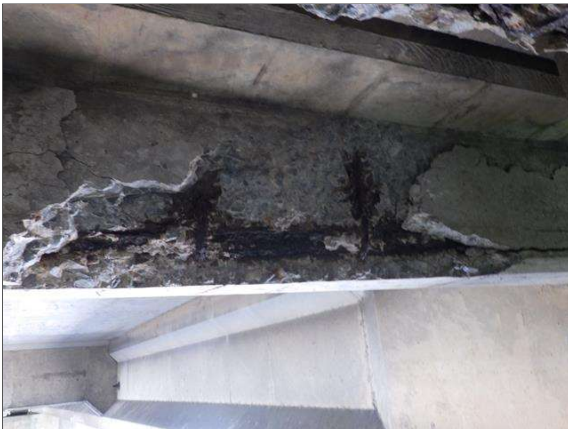
Span 2 Beam 3: DELAMINATED AND SPALLED AREA UP TO FULL LENGTH X FULL WIDTH X FULL HEIGHT WITH EXPOSED REINFORCEMENT IN BAY 3 END DIAPHRAGM AT BENT 1
