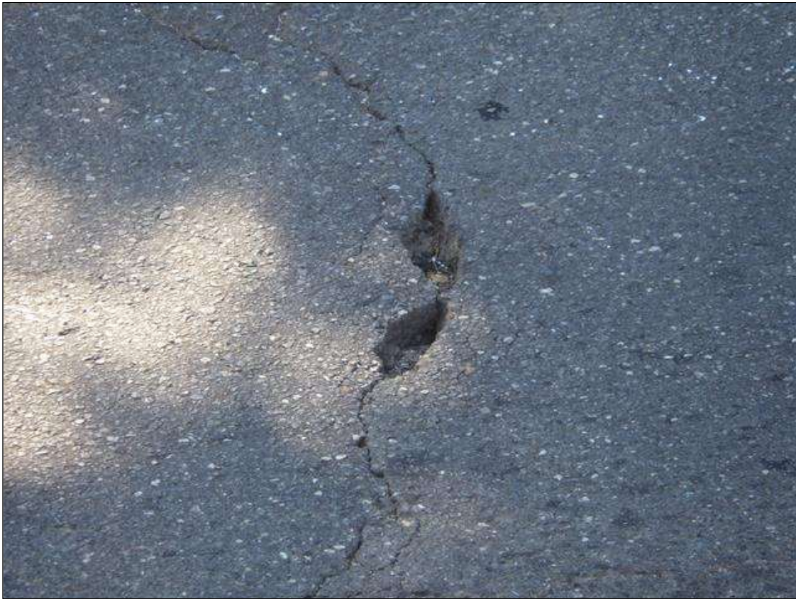
1 FOOT 4 INCHES WIDE X 3 INCHES LONG X 2 INCHES DEEP SPALLED AREA IN THE WEST APPROACH ASPHALT WEARING SURFACE, 8 FEET FROM END BENT 1
