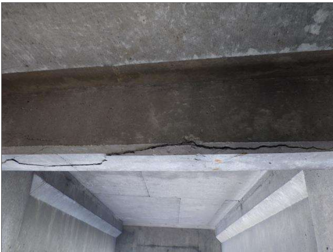
Span 3 Beam 2: DELAMINATED AREA UP TO FULL WIDTH X 10 INCHES LONG X 2 INCHES HIGH IN BAY 2 END DIAPHRAGM AT BENT 3
