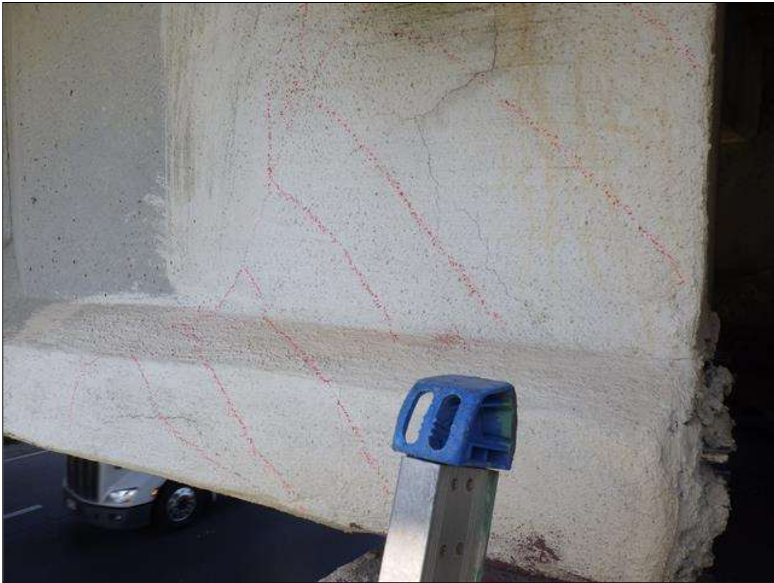
Span 2 Beam 5: DELAMINATED PATCH AREA UP TO 3 FEET 11 INCHES LONG X 2 FEET 5 INCHES HIGH X 9 INCHES WIDE IN THE RIGHT FACE OF THE WEB AND BOTTOM FLANGE AT BENT 2
