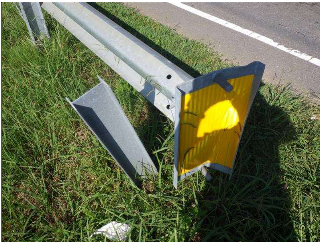
1 FOOT LONG IMPACT DAMAGE TO THE SOUTHEAST GUARDRAIL END TREATMENT WITH THE END POST DETACHED (PRIORITY ACTION REQUEST)
