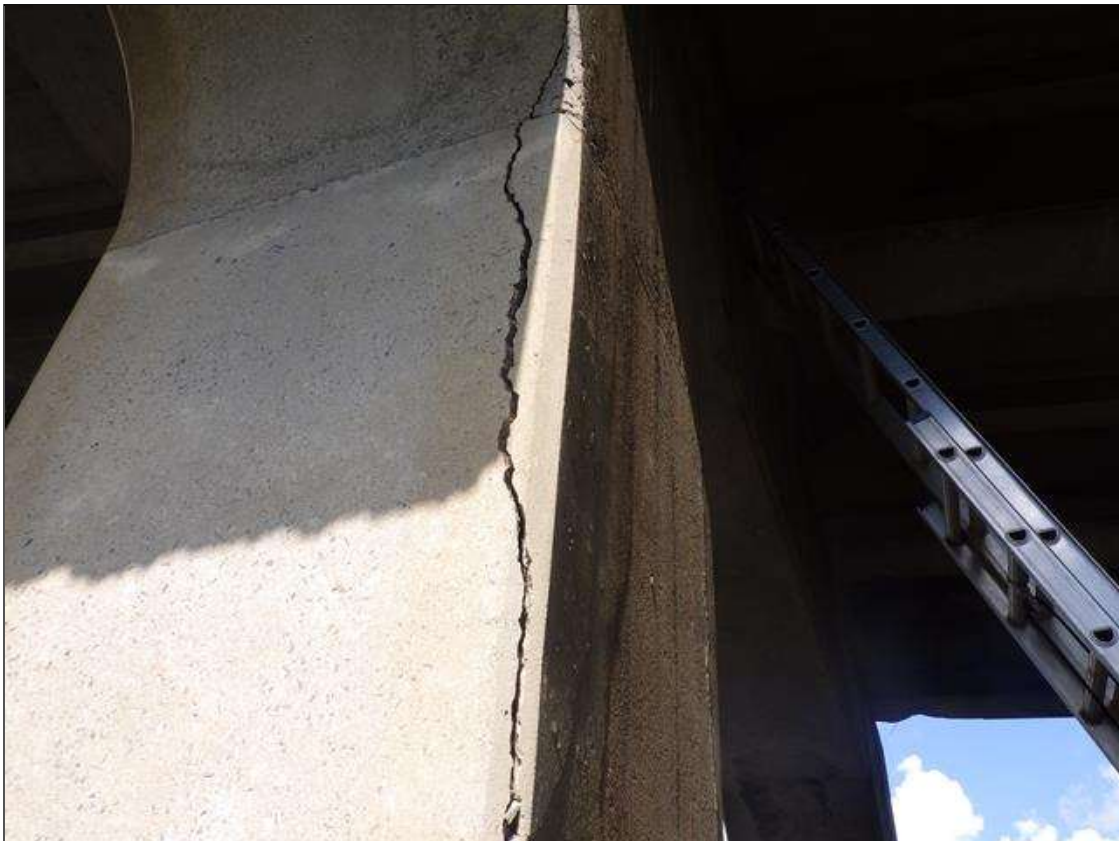
Bent 3 Pile 2: DELAMINATED AND SPALLED AREA UP TO FULL HEIGHT X 11 INCHES LONG X 9 INCHES WIDE WITH EXPOSED REINFORCEMENT IN THE SOUTHEAST CORNER
