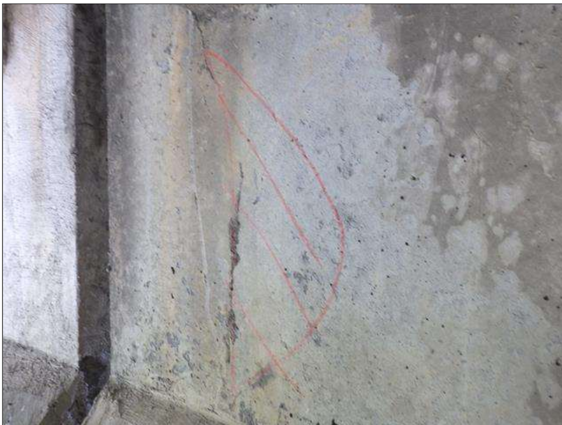
Span 4 Beam 1: DELMINATED AREA UP TO 6 INCHES LONG X 1 FOOT 4 INCHES HIGH IN THE RIGHT WEB, 6 INCHES FROM THE END OF GIRDER AT BENT 3
