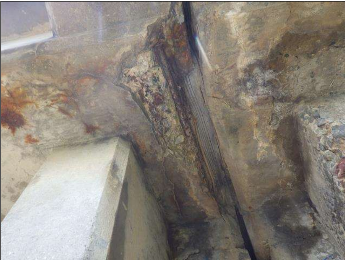
Span 3 Deck: SPALLED AREA UP TO 8 INCHES LONG X 2 FEET WIDE X 4 INCHES DEEP WITH EXPOSED REINFORCEMENT IN THE SOUTH OVERHANG AT BENT 3
