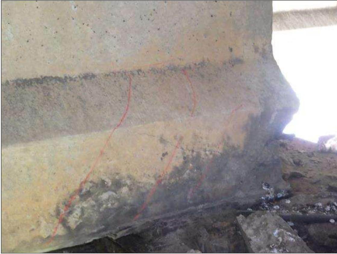
Span 1 Beam 3: 1 FOOT 6 INCHES LONG X 10 INCHES HIGH X 3 INCHES WIDE SPALLED AND DELAMINATED AREA WITH (2) EXPOSED PRESTRESSING STRANDS IN THE RIGHT BOTTOM FLANGE AT BENT 1 (PRIORITY ACTION REQUEST)
