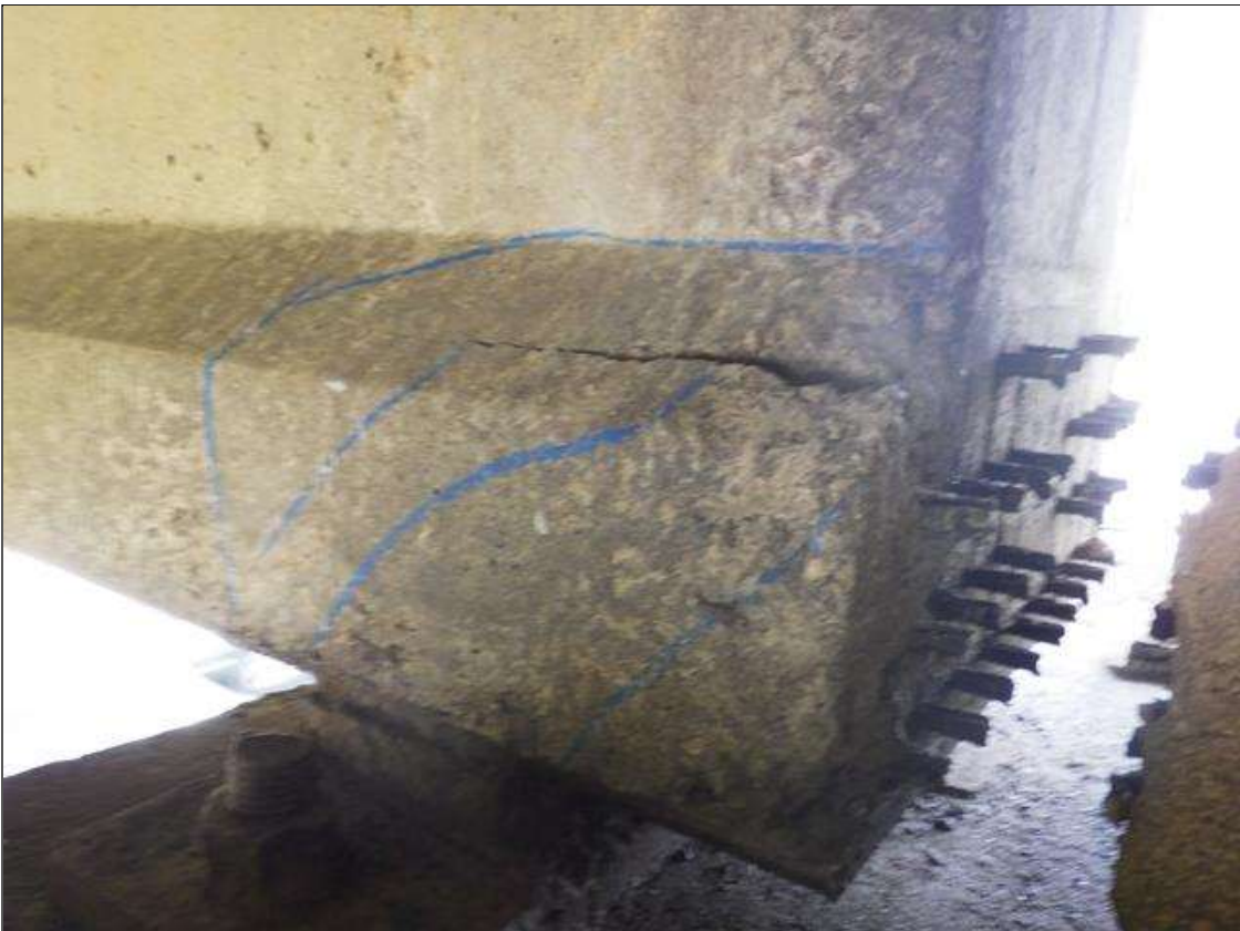
Span 3 Beam 3: PATCHED AREA UP TO 1 FOOT LONG X 10 INCHES HIGH X 3 INCHES WIDE IN THE RIGHT BOTTOM FLANGE AT BENT 2
