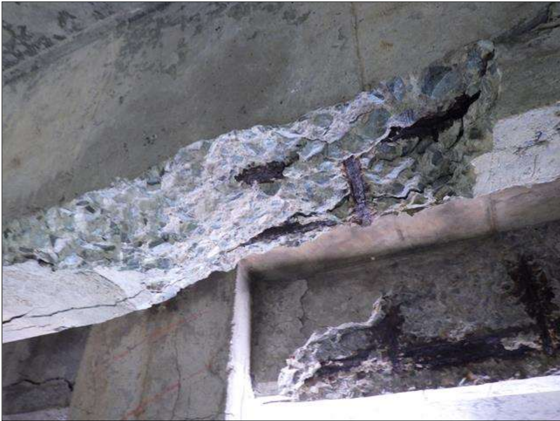
Span 1 Beam 2: DELAMINATED AND SPALLED AREA UP TO FULL LENGTH X FULL WIDTH X FULL HEIGHT WITH EXPOSED REINFORCEMENT IN BAY 2 END DIAPHRAGM AT BENT 1
