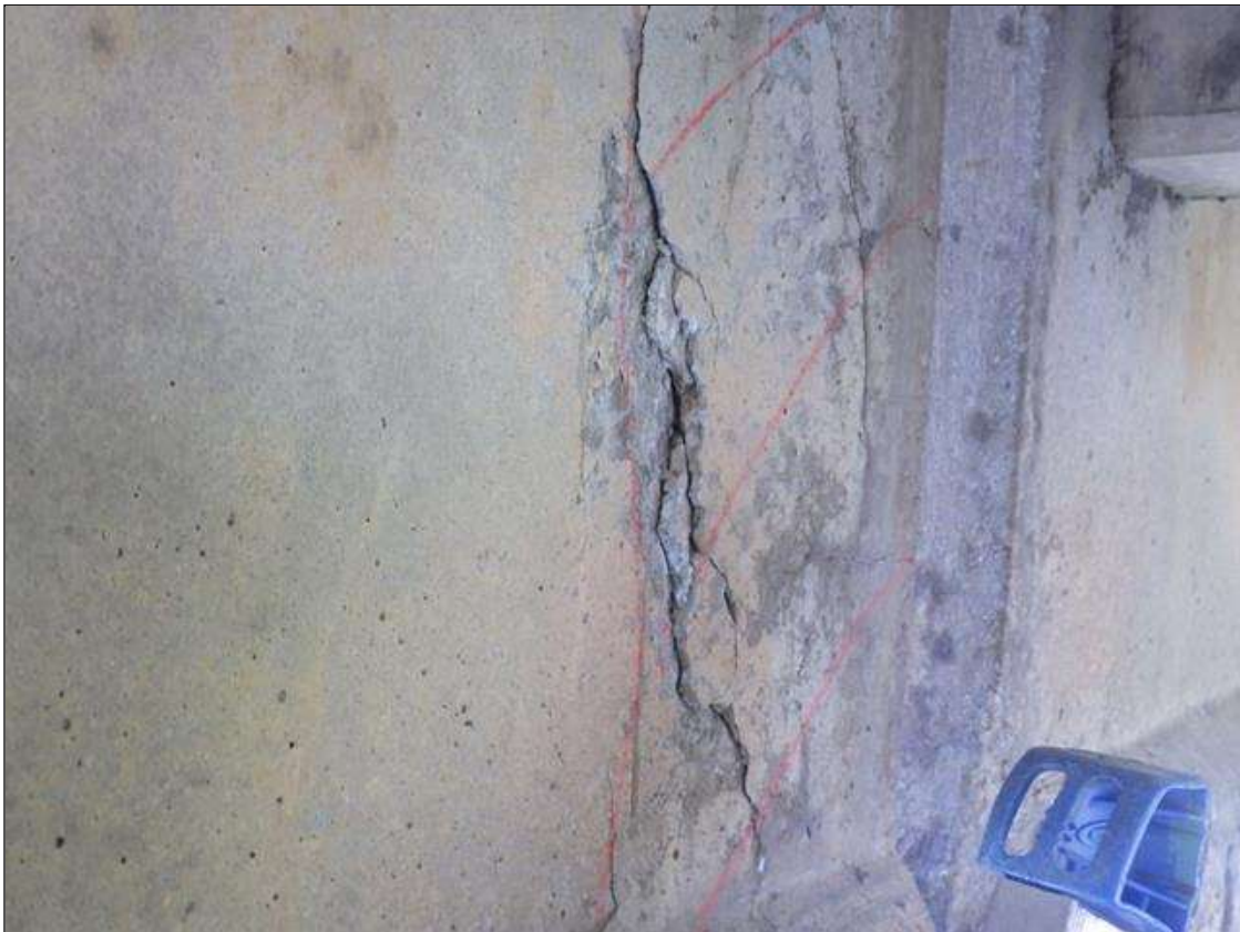
Span 3 Beam 4: DELAMINATED AND SPALLED AREA UP TO 1 FOOT 2 INCHES LONG X FULL HEIGHT X 1 INCH DEEP IN THE LEFT FACE OF THE WEB AT BENT 2
