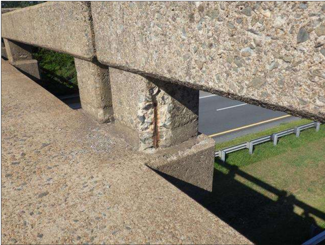
Span 3 Left Bridge Rail: (2) SPALLS UP TO 7 INCHES HIGH X 3 INCHES LONG X 1 INCH WIDE WITH EXPOSED REINFORCEMENT, (1) IN POST 1 AND (1) IN POST 4 (POST 4 SHOWN)
