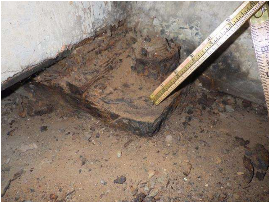
Span 4 Far Bearing: ACTIVE CORROSION THROUGHOUT THE GIRDER 1 BEARING WITH 1/16 INCH SECTION LOSS (LESS THAN 25 PERCENT SECTION LOSS)
