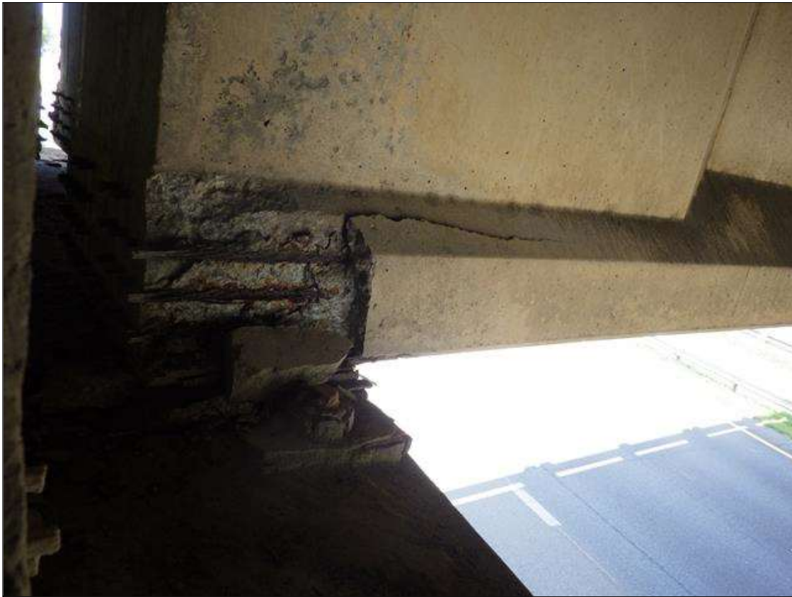
Span 2 Beam 2: 2 FEET 6 INCHES LONG X 10 INCHES HIGH X 3 INCHES WIDE SPALLED AREA WITH (3) EXPOSED PRESTRESSING STRANDS IN THE RIGHT BOTTOM FLANGE AT BENT 1 (PRIORITY ACTION REQUEST)
