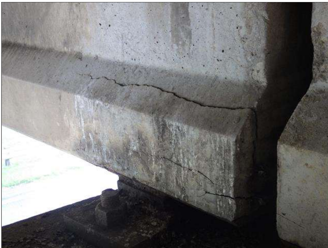
Span 3 Beam 2: DELAMINATED AREA UP TO 2 FEET LONG X 9 INCHES HIGH X 2 INCHES WIDE IN THE RIGHT BOTTOM FLANGE AT BENT 3
