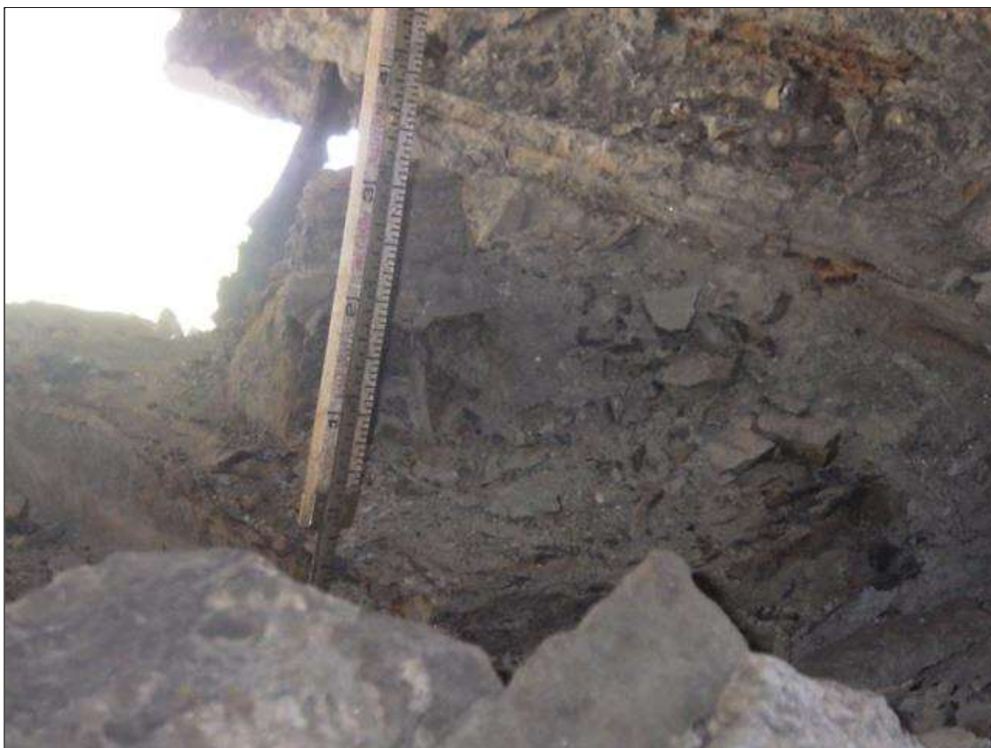
Span 2 Beam 5 - Near Bearing: ACTIVE CORROSION UP TO FULL PERIMETER X FULL HEIGHT WITH 1/16 INCH SECTION LOSS THROUGHOUT GIRDER 5 BEARING
