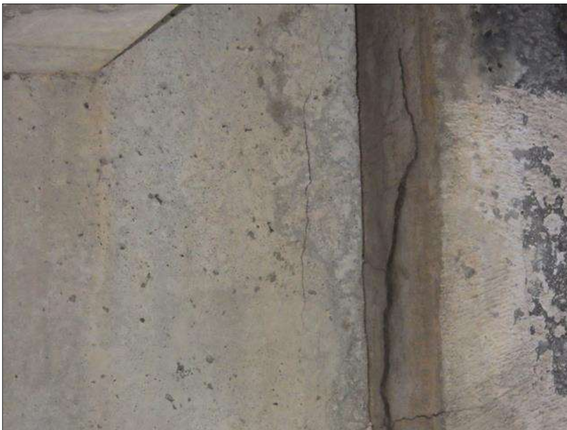
Span 4 Beam 4: VERTICAL CRACK UP TO 1 FOOT HIGH X 1/32 INCH WIDE IN THE LEFT WEB, 2 INCHES FROM END OF GIRDER AT BENT 3
