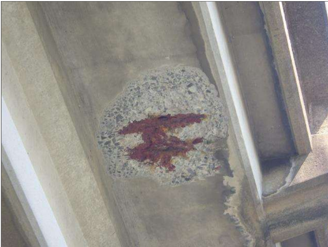
Span 3 Deck: SPALLED AREA UP TO 2 FEET DIAMETER X 2 INCHES DEEP WITH PAINTED EXPOSED REINFORCEMENT IN THE UNDERSIDE OF THE SOUTH OVERHANG ABOVE THE LEFT NORTHBOUND LANE
