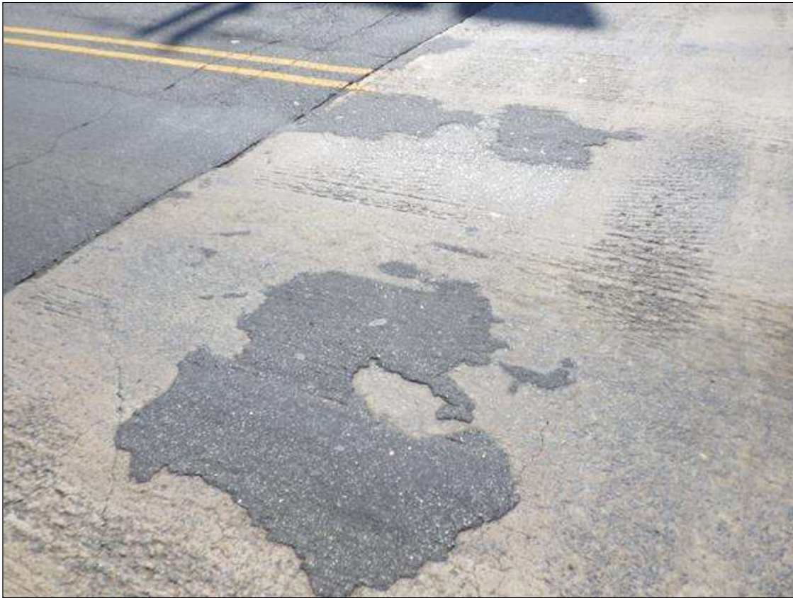
Span 4 Deck: (3) PATCHED AREAS UP TO 4 FEET 3 INCHES LONG X 4 FEET 8 INCHES WIDE IN THE WESTBOUND LANE AT END BENT 2
