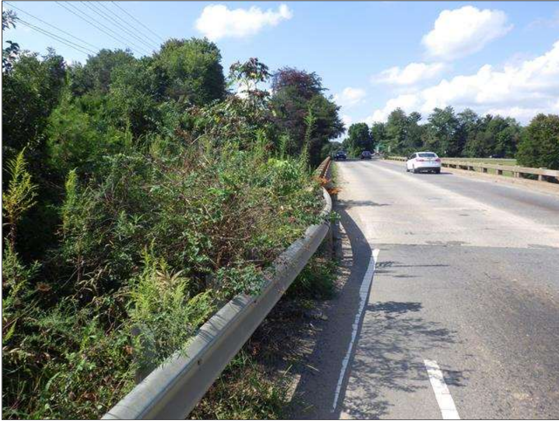
SOUTHEAST DELINEATOR IS MISSING (PRIORITY ACTION REQUEST)
