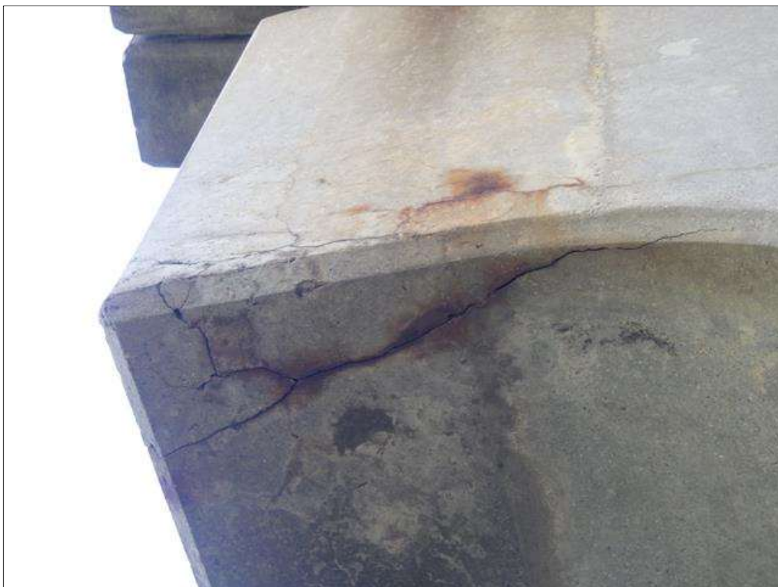
Bent 3 Cap 1: DELAMINATED AREA UP TO 2 FEET LONG X 1 FOOT HIGH X 8 INCHES WIDE WITH RUST STAINING IN THE WEST FACE AND UNDERSIDE AT THE SOUTH END
