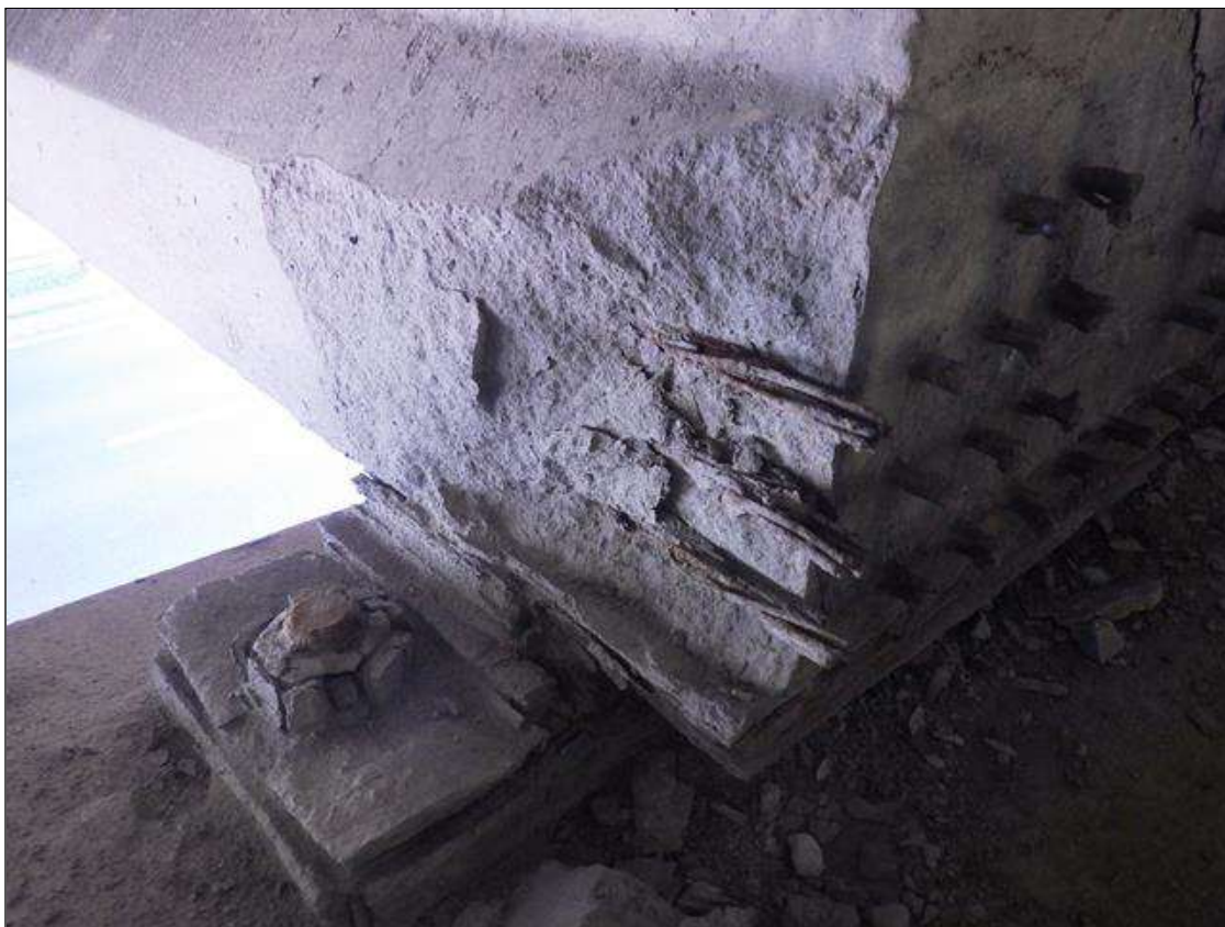
Span 2 Beam 3: 1 FEET 2 INCHES LONG X 10 INCHES HIGH X 2 INCHES WIDE SPALLED AREA WITH (2) EXPOSED PRESTRESSING STRANDS IN THE LEFT BOTTOM FLANGE AT BENT 1 (PRIORITY ACTION REQUEST)
