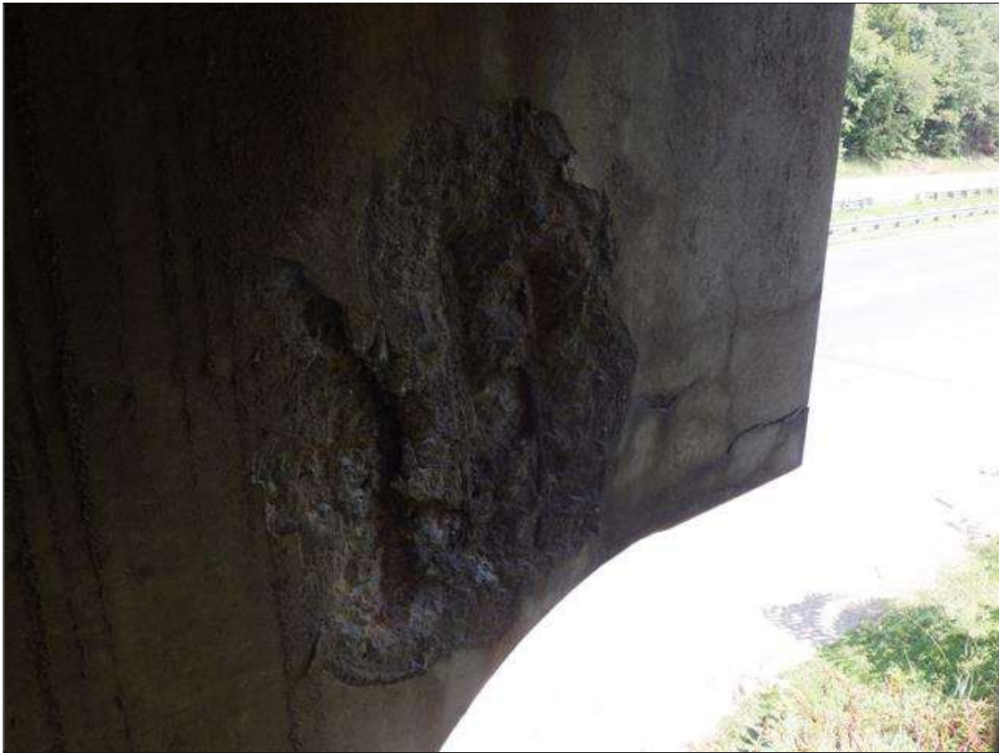
Bent 1 Cap 1: DELAMINATED AND SPALLED AREA UP TO 3 FEET 7 INCHES LONG X 2 FEET 3 INCHES HIGH X 2 INCH DEEP WITH EXPOSED REINFORCEMENT IN THE WEST FACE BELOW GIRDER 4
