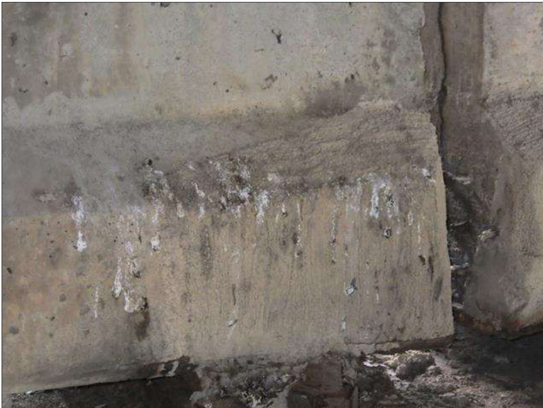
Span 4 Beam 4: PATCHED AREA UP TO 1 FOOT LONG X 10 INCHES HIGH X 5 INCHES WIDE IN THE LEFT BOTTOM FLANGE AT BENT 3
