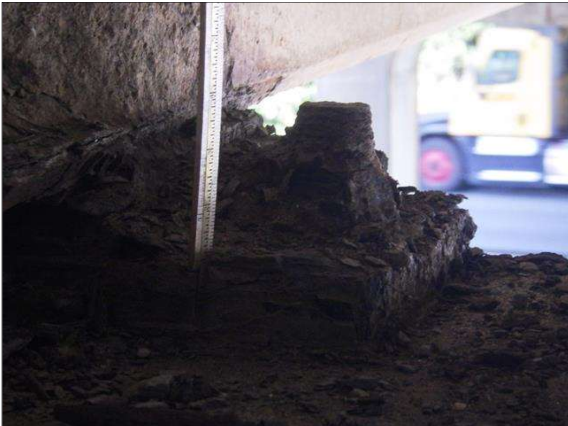
Span 1 Beam 4 - Far Bearing: ACTIVE CORROSION UP TO FULL PERIMETER X FULL HEIGHT WITH 1/16 INCH SECTION LOSS THROUGHOUT GIRDER 4 BEARING
