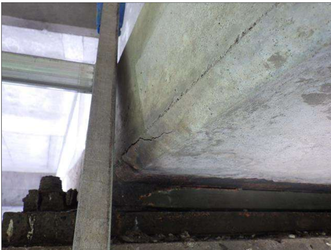
Span 4 Beam 3: LONGITUDINAL CRACK UP TO 6 INCHES LONG X 1/16 INCH WIDE IN THE RIGHT BOTTOM FLANGE ADJACENT TO THE EMBEDDED PLATE AT BENT 3
