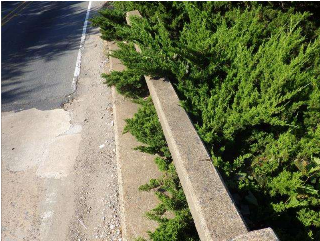
25 FEET LONG X 3 FEET HIGH X 2 FEET WIDE VEGETATION GROWTH THROUGH THE NORTH BRIDGE RAIL AT END BENT 1
