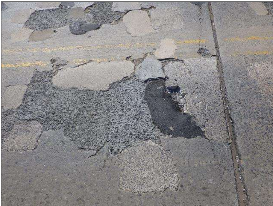
Span 2 Deck: 6 FEET 7 INCHES LONG X 4 FEET WIDE SPALLED AND DELAMINATED PATCHED AREA WITH EXPOSED REINFORCEMENT IN THE WESTBOUND LANE AT BENT 1 (PRIORITY ACTION REQUEST)
