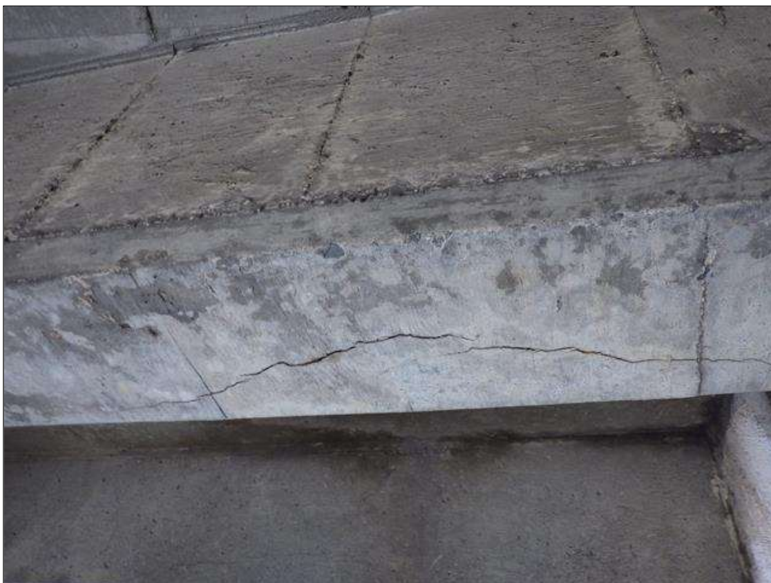
Span 4 Beam 1: LONGITUDINAL CRACK UP TO INTERMITTENT FULL WIDTH X 1/16 INCH WIDE IN BAY 1 END DIAPHRAGM AT BENT 3
