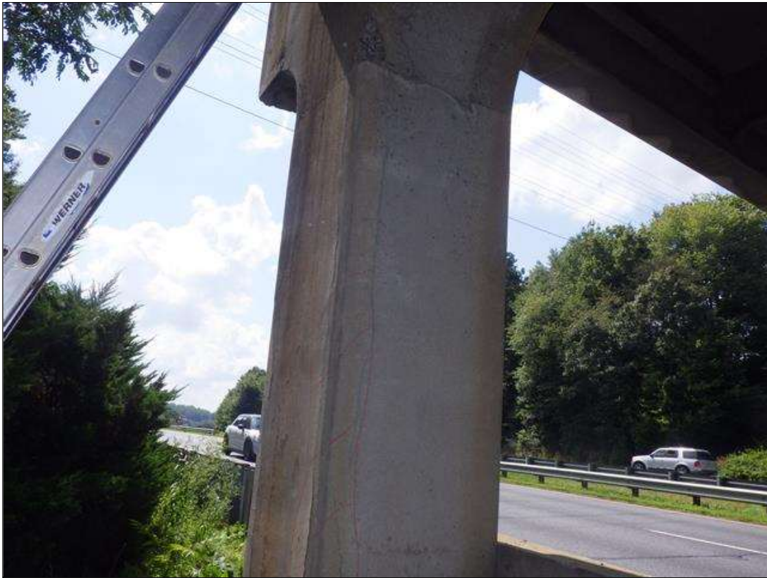
Bent 3 Pile 2: DELAMINATED AND SPALLED AREA UP TO FULL HEIGHT X 11 INCHES LONG X 9 INCHES WIDE IN THE NORTHEAST CORNER
