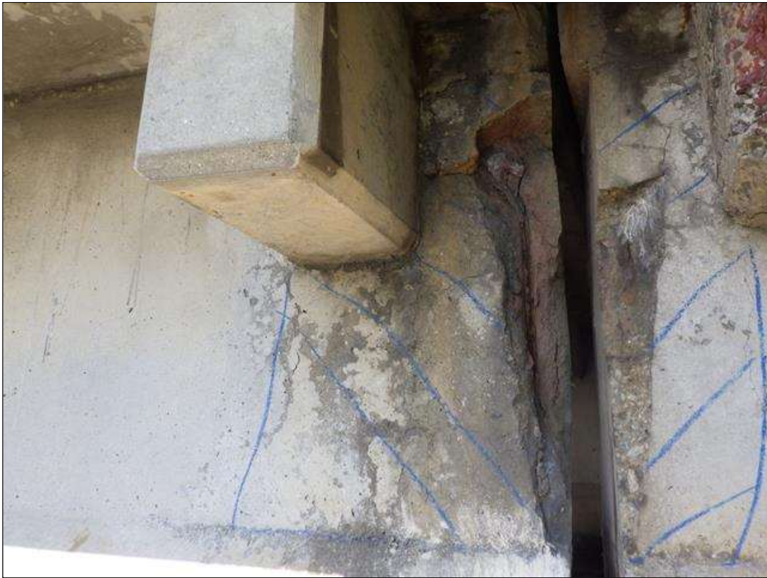
Span 3 Beam 4: DELAMINATED AND SPALLED AREA UP TO 1 FOOT 9 INCHES LONG X FULL HEIGHT X FULL WIDTH IN THE RIGHT SIDE OF THE WEB AND EAST FACE WITH EXPOSED EMBEDDED PLATE AT BENT 3
