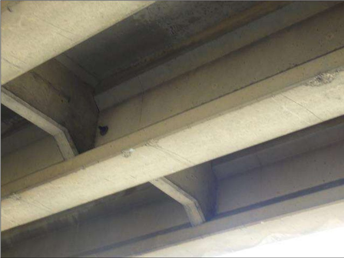
Span 2 Beam 4: (4) SPALLED AREAS UP TO 10 INCHES LONG X 4 INCHES WIDE X 2 INCHES HIGH IN THE LEFT BOTTOM FLANGE ABOVE THE RIGHT SOUTHBOUND THRU LANE
