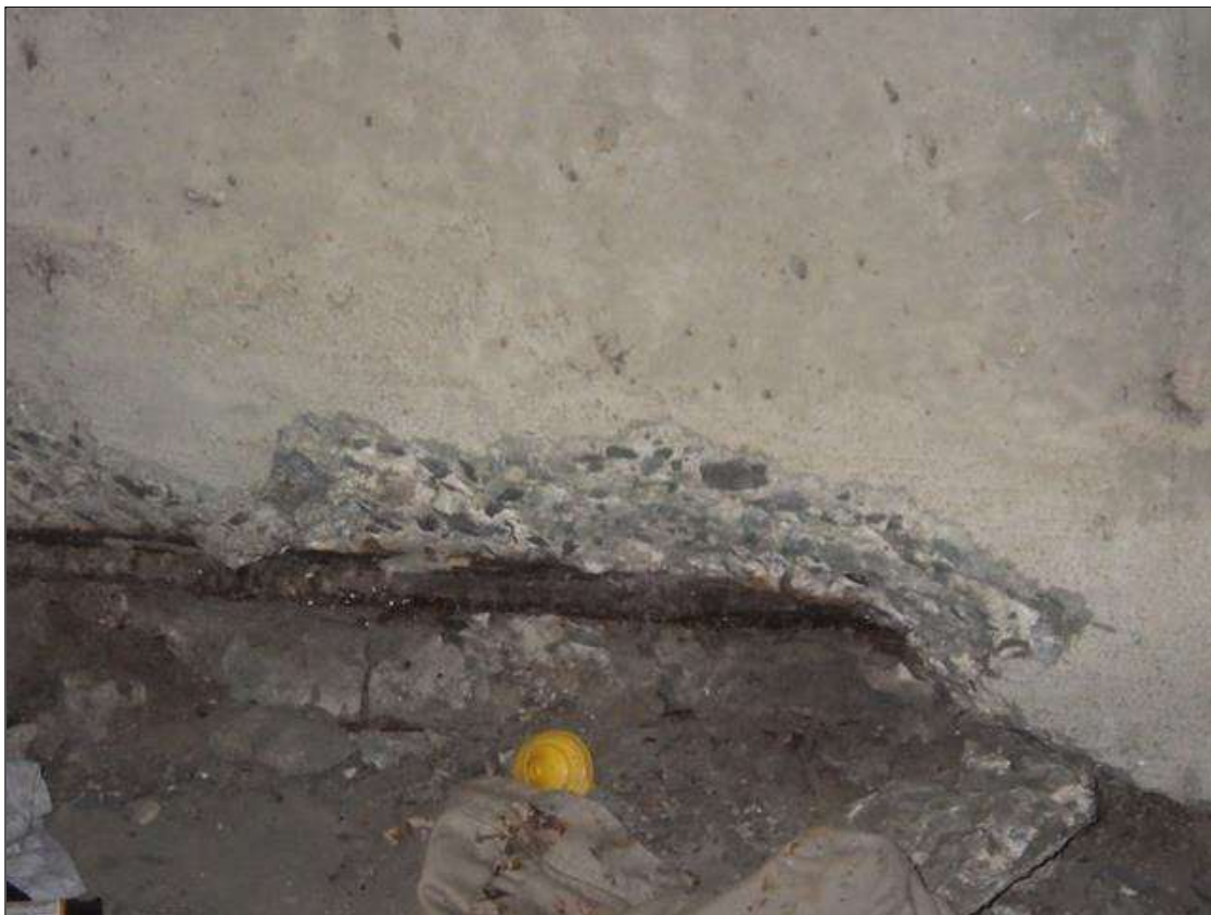
End Bent 1 Abutment: SPALLED AREA UP TO 2 FEET LONG X 6 INCHES HIGH X 3 INCHES DEEP WITH EXPOSED REINFORCEMENT IN BAY 1
