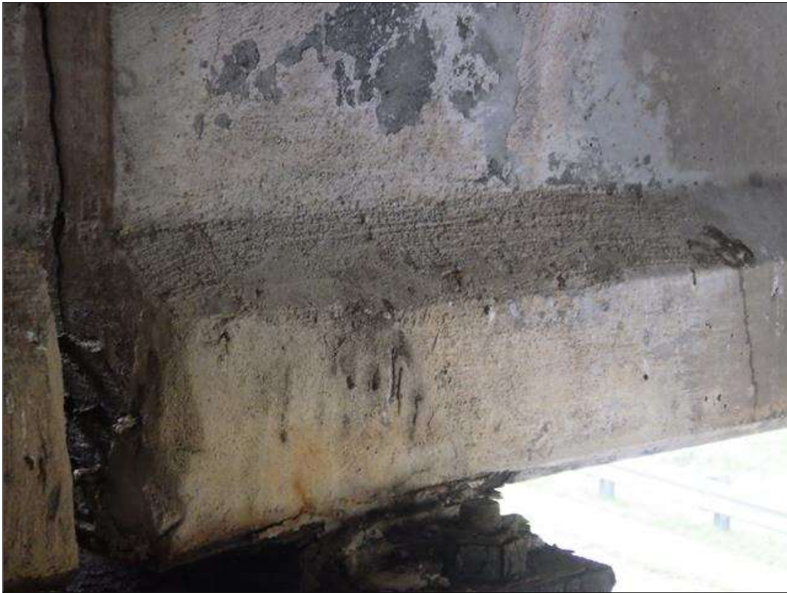
Span 3 Beam 4: PATCHED AREA UP TO 2 FEET LONG X 10 INCHES HIGH X 3 INCHES WIDE IN THE LEFT BOTTOM FLANGE AT BENT 3
