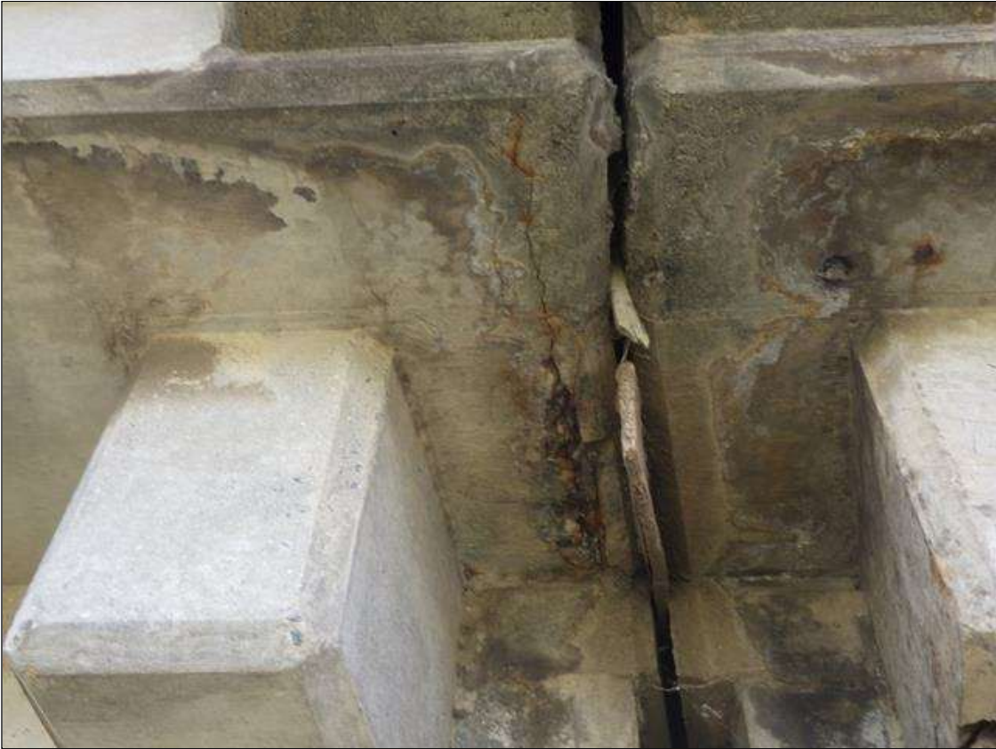
Span 3 Deck: DELAMINATED AND SPALLED AREA UP TO 3 INCHES LONG X 2 FEET WIDE X 1 INCH DEEP WITH EXPOSED REINFORCEMENT IN THE UNDERSIDE OF THE NORTH OVERHANG AT BENT 2
