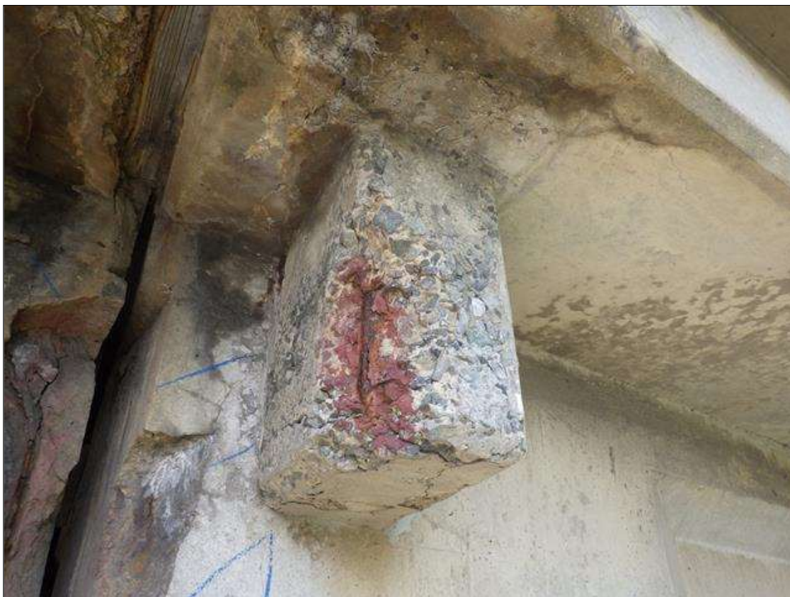
Span 4 Beam 4: DELAMINATED AND SPALLED AREA UP TO FULL LENGTH X FULL WIDTH X FULL HEIGHT WITH EXPOSED REINFORCEMENT IN THE SOUTH OVERHANG END DIAPHRAGM AT BENT 3
