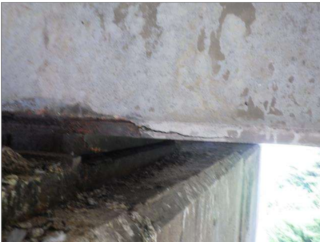
Span 4 Beam 2: LONGITUDINAL CRACKS UP TO 6 INCHES LONG X 1/16 INCH WIDE IN THE RIGHT BOTTOM FLANGE AND LEFT BOTTOM FLANGE ADJACENT TO THE EMBEDDED PLATE AT BENT 3
