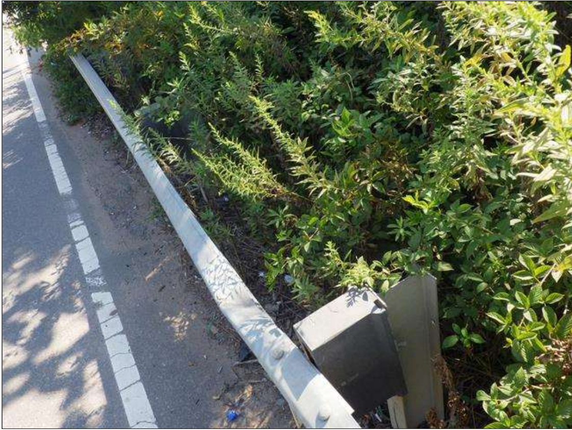
7 FEET LONG AREA OF IMPACT DAMAGE TO THE SOUTHEAST GUARDRAIL WITH POST 8 DETACHED, 30 FEET FROM END BENT 2 (PRIORITY ACTION REQUEST)
