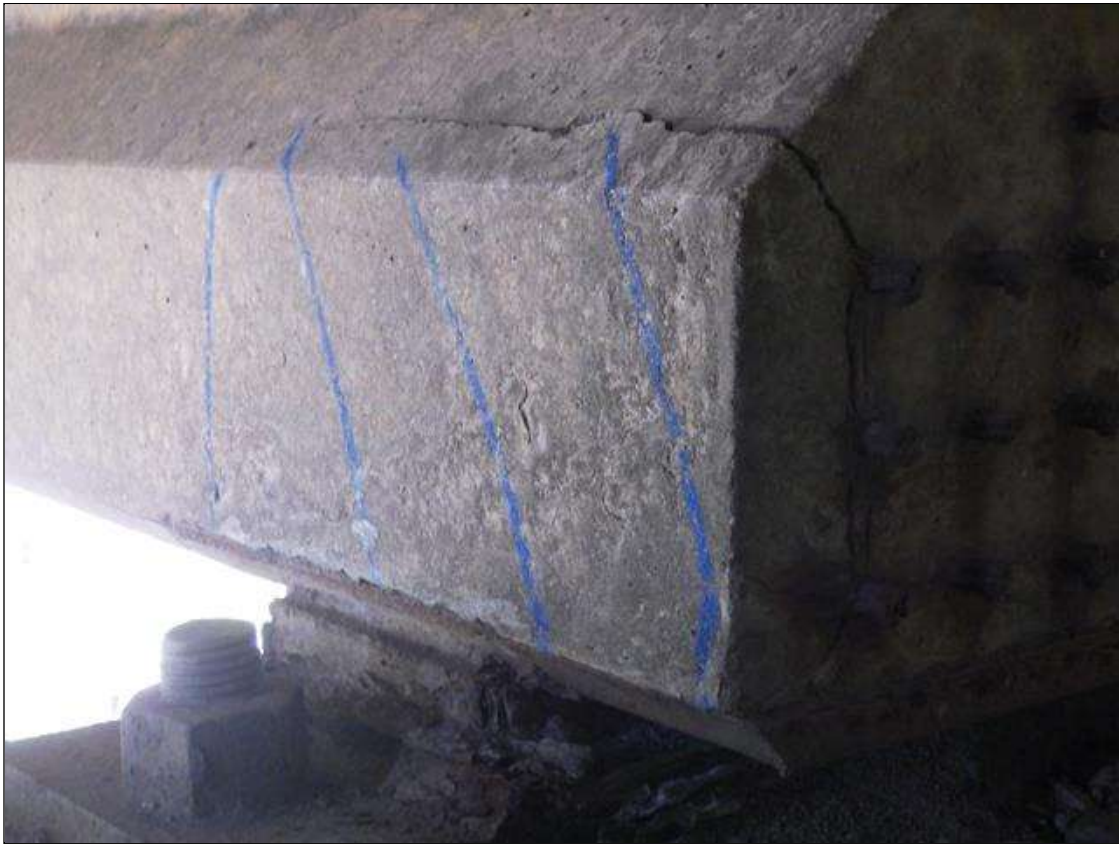
Span 1 Beam 2: DELAMINATED AREA UP TO 1 FOOT 4 INCHES LONG X 7 INCHES HIGH X 2 INCHES WIDE IN THE LEFT BOTTOM FLANGE AT BENT 1
