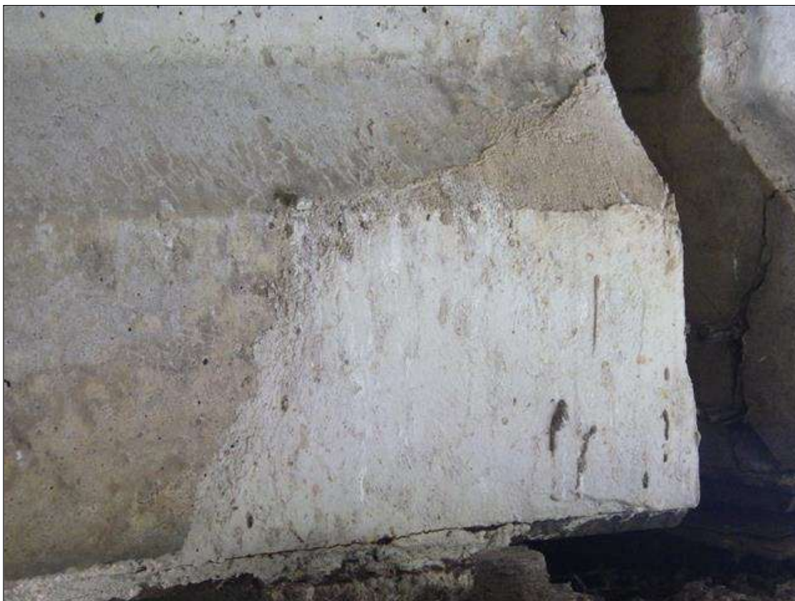
Span 4 Beam 3: PATCHED AREA UP TO 1 FOOT LONG X 10 INCHES HIGH X 3 INCHES WIDE IN THE LEFT BOTTOM FLANGE AT BENT 3
