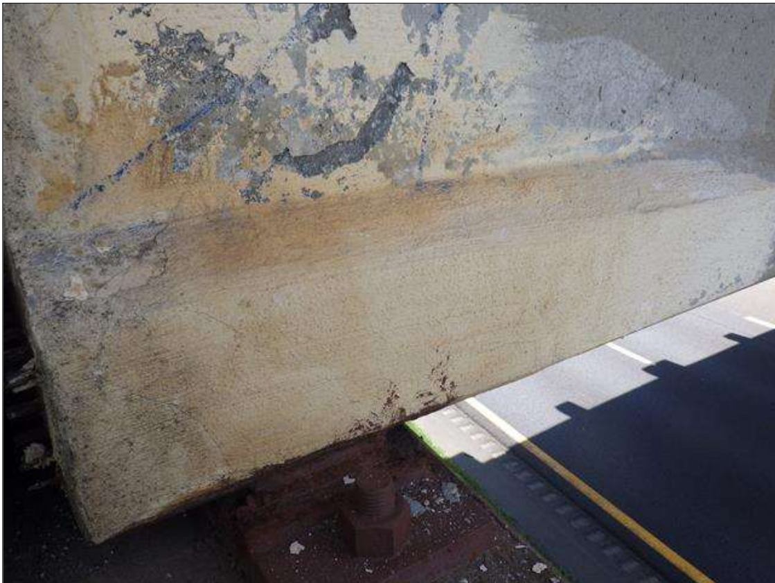
Span 2 Beam 1: PATCHED AREA UP TO 3 FEET 5 INCHES LONG X 8 INCHES HIGH X 3 INCHES WIDE IN THE LEFT BOTTOM FLANGE AT BENT 2
