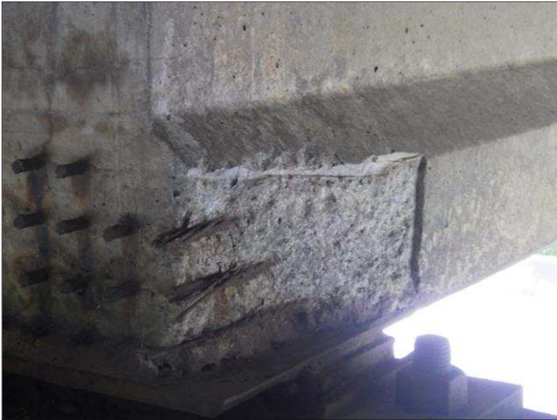
Span 2 Beam 2: 1 FOOT 3 INCHES LONG X 8 INCHES HIGH X 4 INCHES WIDE SPALLED AREA WITH (3) EXPOSED PRESTRESSING STRANDS IN THE LEFT BOTTOM FLANGE AT BENT 2 (PRIORITY ACTION REQUEST)
