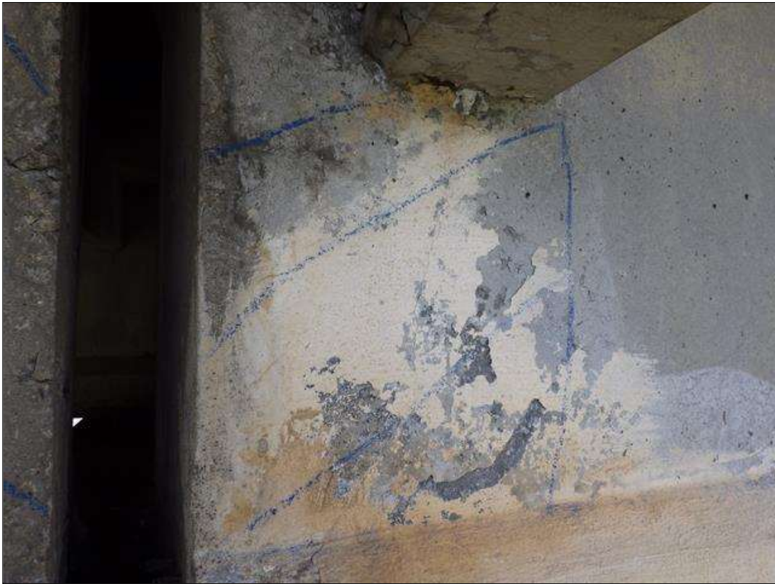
Span 2 Beam 1: DELAMINATED AREA UP TO 1 FOOT 5 INCHES LONG X FULL HEIGHT X FULL WIDTH IN THE LEFT SIDE OF THE WEB AT BENT 2
