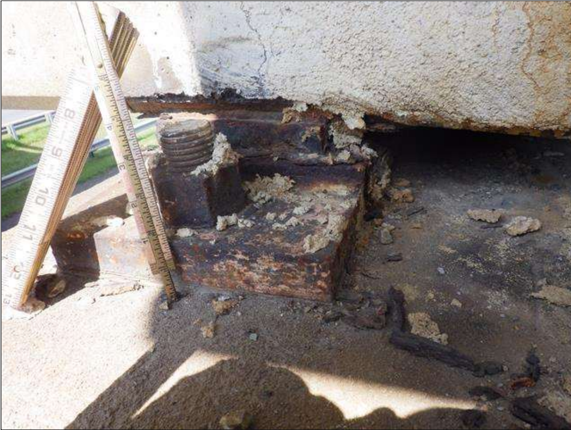
Span 3 Beam 4 - Far Bearing: ACTIVE CORROSION THROUGHOUT THE GIRDER 4 BEARING WITH 1/32 INCH SECTION LOSS
