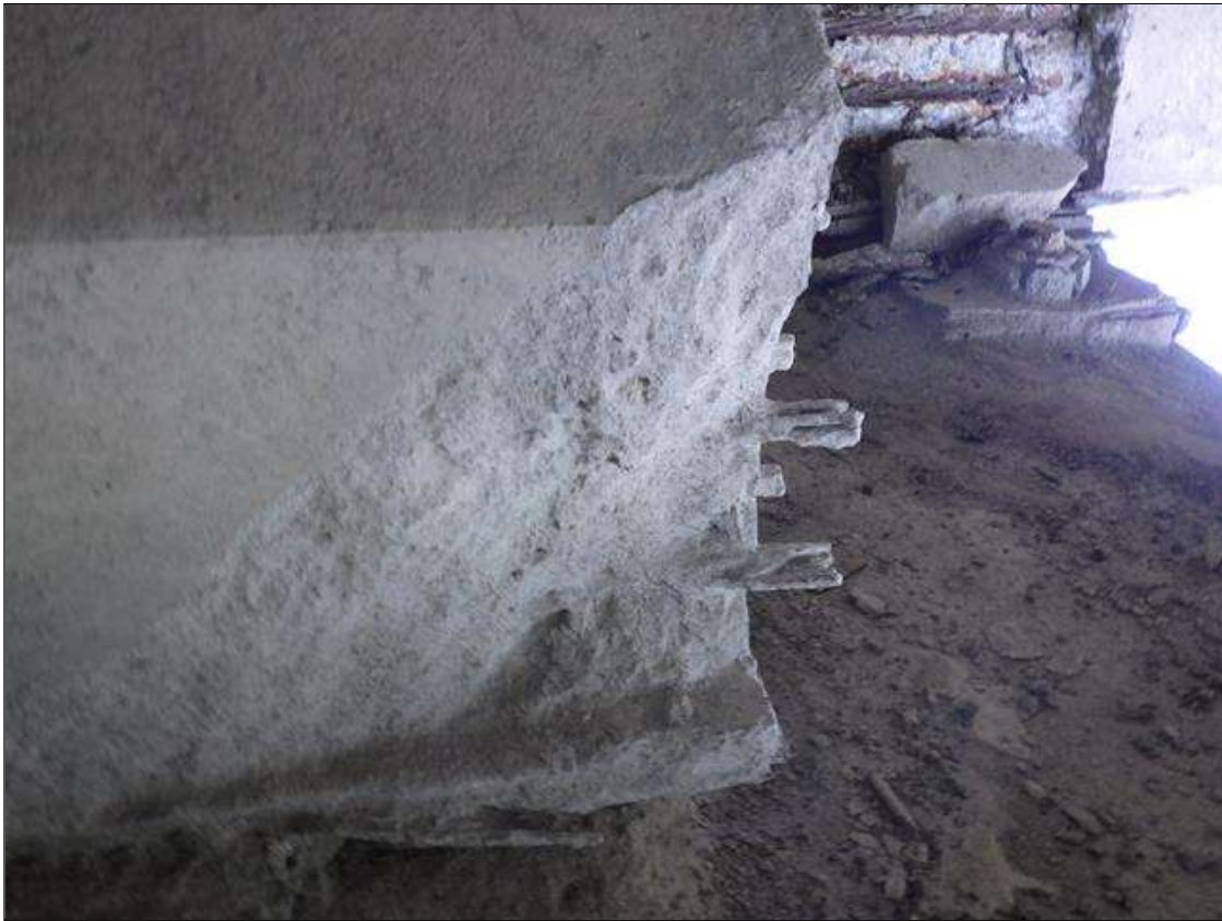
Span 1 Beam 2: 9 INCHES LONG X 7 INCHES HIGH X 4 INCHES WIDE SPALLED AREA WITH (2) EXPOSED PRESTRESSING STRANDS IN THE RIGHT BOTTOM FLANGE AT BENT 1 (PRIORITY ACTION REQUEST)
