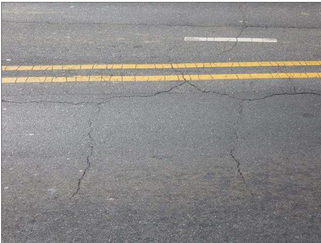
GREATER THAN 50 FEET LONG X INTERMITTENT FULL WIDTH MAP CRACKING UP TO 1/4 INCH WIDE IN THE EAST APPROACH ASPHALT WEARING SURFACE AT END BENT 2 (WEST APPROACH SIMILAR)
