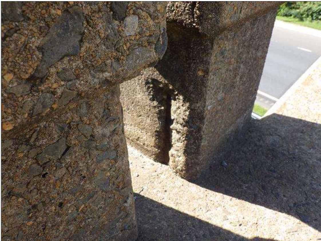
Span 3 Right Bridge Rail: (2) SPALLS UP TO 8 INCHES HIGH X 1 INCH WIDE X 1/2 INCH DEEP WITH EXPOSED REINFORCEMENT, (1) IN POST 3 AND (1) IN POST 4
