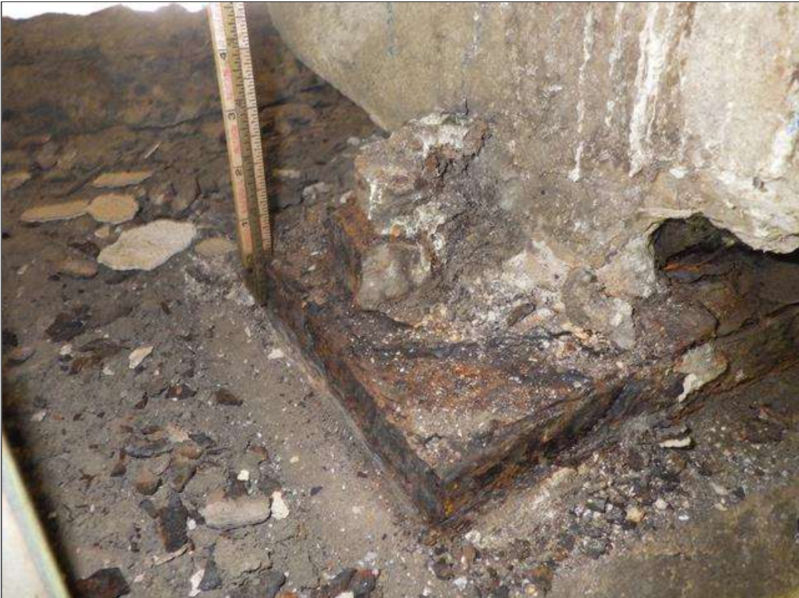
Span 1 Beam 3 - Far Bearing: ACTIVE CORROSION UP TO FULL PERIMETER X FULL HEIGHT WITH 1/16 INCH SECTION LOSS THROUGHOUT GIRDER 3 BEARING
