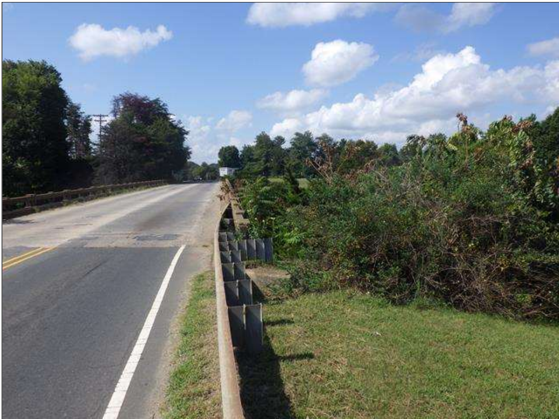
NORTHEAST DELINEATOR IS MISSING (PRIORITY ACTION REQUEST)
