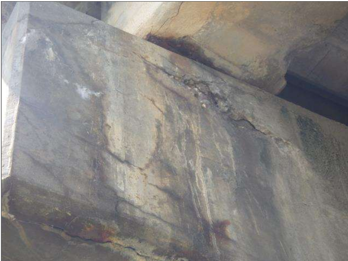
Bent 1 Cap 1: DELAMINATED AND SPALLED AREA UP TO 3 FEET LONG X FULL HEIGHT X FULL WIDTH WITH EXPOSED REINFORCEMENT AND EFFLORESCENCE IN THE EAST AND SOUTH FACES
