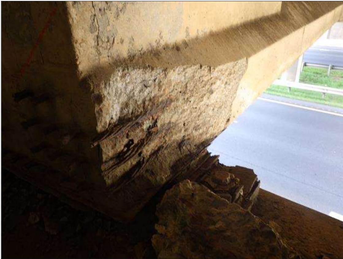
Span 2 Beam 3: 1 FEET 9 INCHES LONG X 10 INCHES HIGH X 2 INCHES WIDE SPALLED AREA WITH (3) EXPOSED PRESTRESSING STRANDS IN THE RIGHT BOTTOM FLANGE AT BENT 1 (PRIORITY ACTION REQUEST)
