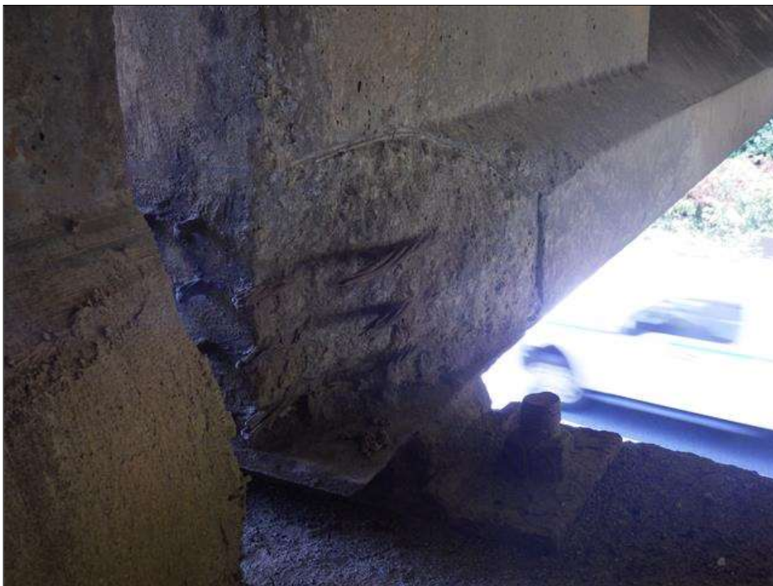
Span 2 Beam 5: 1 FOOT 4 INCHES LONG X 10 INCHES HIGH X 4 INCHES WIDE SPALLED AREA WITH (6) EXPOSED PRESTRESSING STRANDS IN THE LEFT BOTTOM FLANGE AT BENT 2 (PRIORITY ACTION REQUEST)
