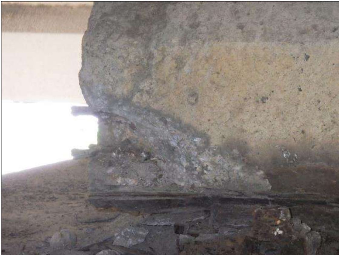
Span 1 Beam 2: 9 INCHES LONG X 4 INCHES HIGH X 3 INCHES WIDE SPALLED AREA WITH (2) EXPOSED PRESTRESSING STRANDS IN THE LEFT BOTTOM FLANGE AT BENT 1 (PRIORITY ACTION REQUEST)
