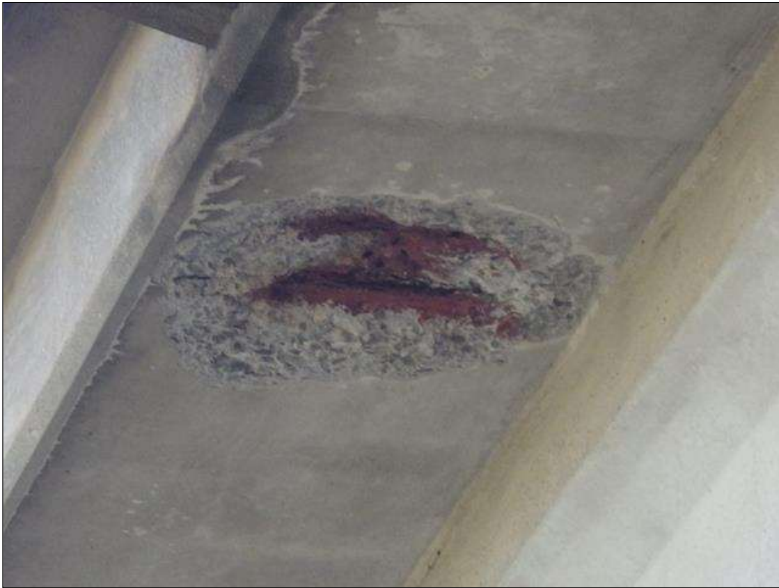
Span 3 Deck: SPALLED AREA UP TO 2 FEET DIAMETER X 2 INCHES DEEP WITH PAINTED EXPOSED REINFORCEMENT IN THE UNDERSIDE OF THE NORTH OVERHANG ABOVE THE RIGHT NORTHBOUND LANE
