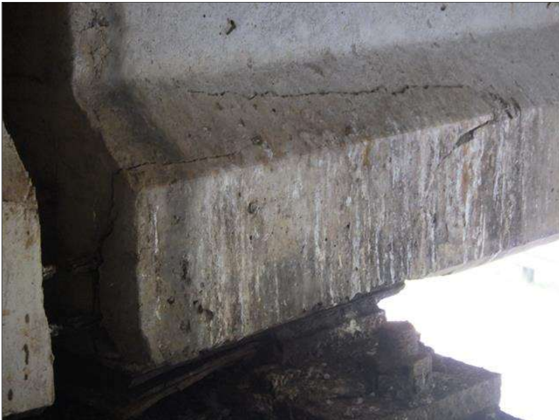
Span 3 Beam 3: DELAMINATED AREA UP TO 2 FEET 1 INCH LONG X 10 INCHES HIGH X 3 INCHES WIDE IN THE LEFT BOTTOM FLANGE AT BENT 3
