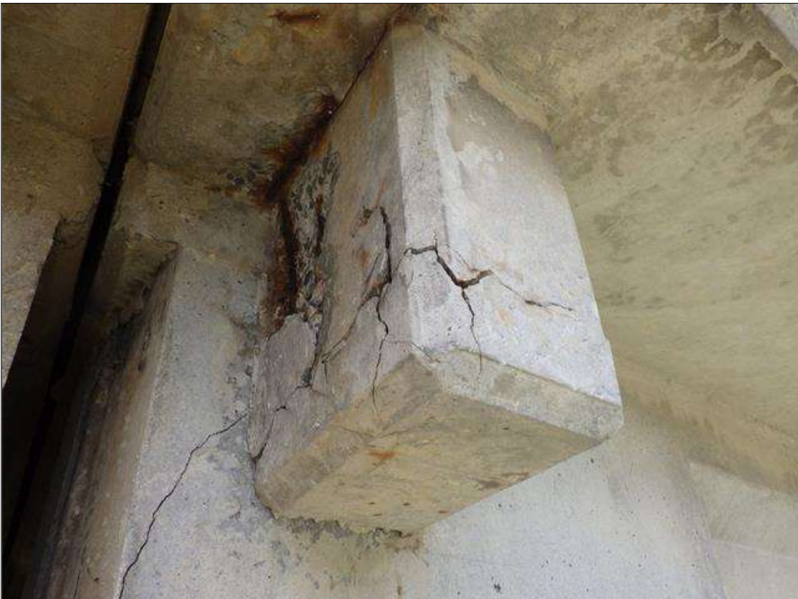
Span 3 Beam 4: DELAMINATED AND SPALLED AREA UP TO FULL LENGTH X FULL WIDTH X FULL HEIGHT WITH EXPOSED REINFORCEMENT IN THE END DIAPHRAGM BELOW THE SOUTH OVERHANG AT BENT 2
