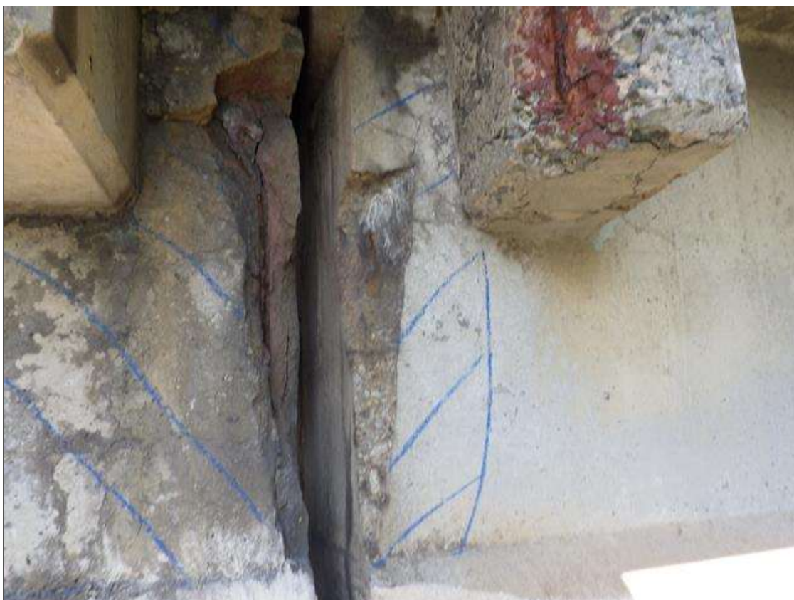
Span 4 Beam 4: DELAMINATED AND SPALLED AREA UP TO 8 INCHES LONG X FULL HEIGHT X 3 INCHES WIDE IN THE RIGHT SIDE OF THE WEB AT BENT 3
