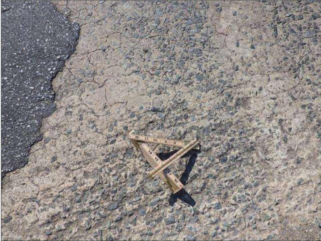
Span 4 Deck: FULL LENGTH X FULL WIDTH MAP CRACKING UP TO 1/16 INCH WIDE THROUGHOUT THE TOP OF THE DECK WITH EXPOSED SURFACE COARSE AGGREGATE (OTHERS SIMILAR)
