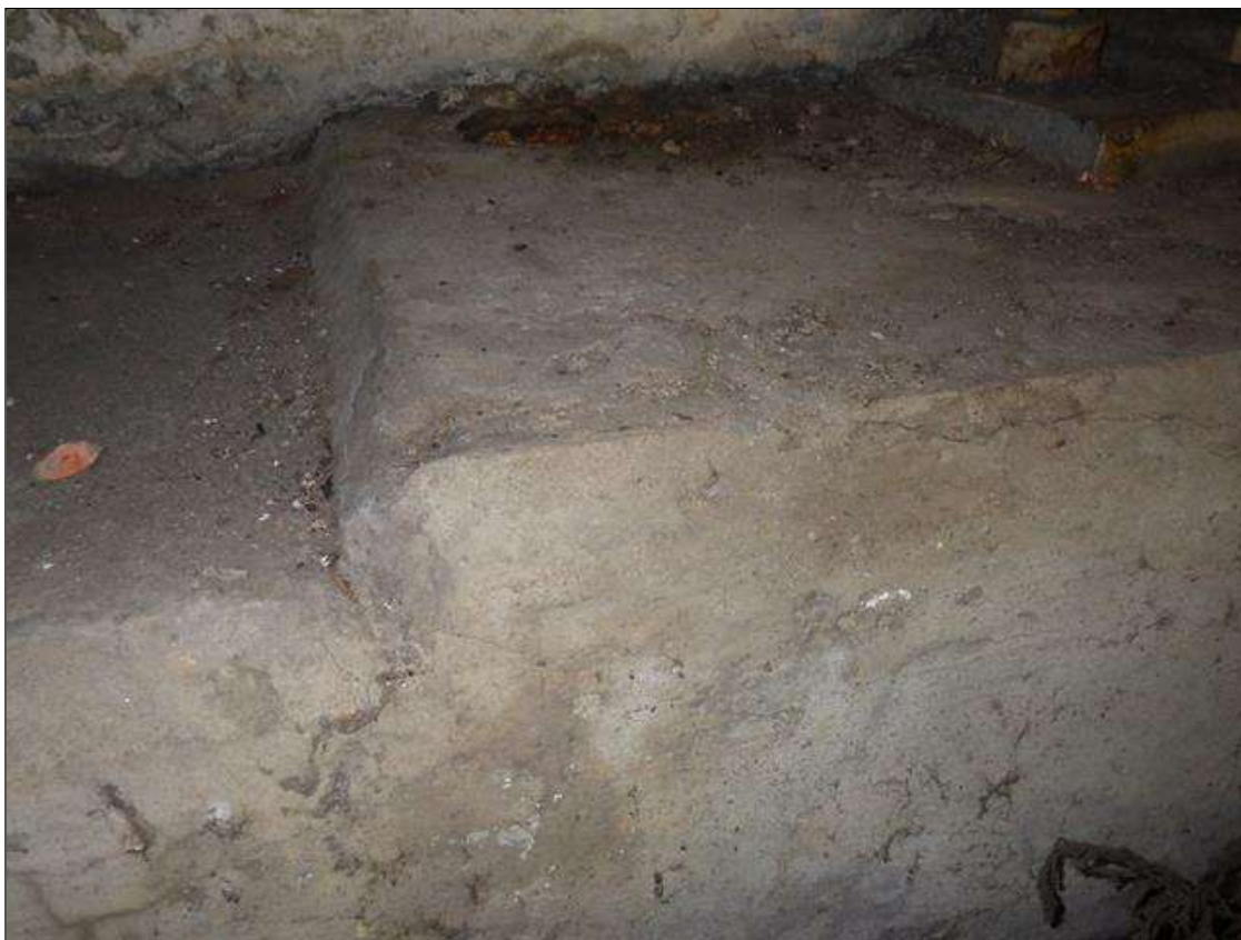
End Bent 2 Cap 1: (2) 7 FEET LONG X 1/16 INCH WIDE LONGITUDINAL CRACKS IN THE CAP BELOW BAY 1
