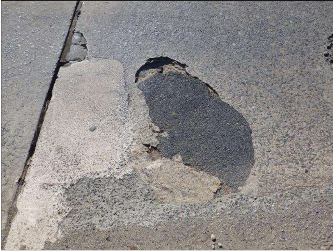
Span 2 Deck: INTERMITTENT FULL LENGTH X INTERMITTENT FULL WIDTH X UP TO 1 1/2 INCHES DEEP DELAMINATIONS, SPALLS, AND FAILED PATCHES THROUGHOUT THE DECK WITH 30 PERCENT OF DECK AREA AFFECTED
