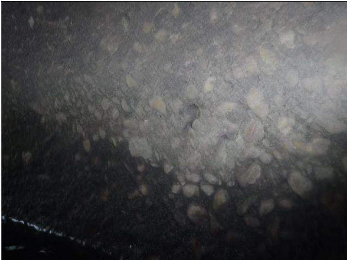
COARSE AGGREGATE EXPOSED ON BARREL WALL (ALL BARRELS SIMILIAR)
