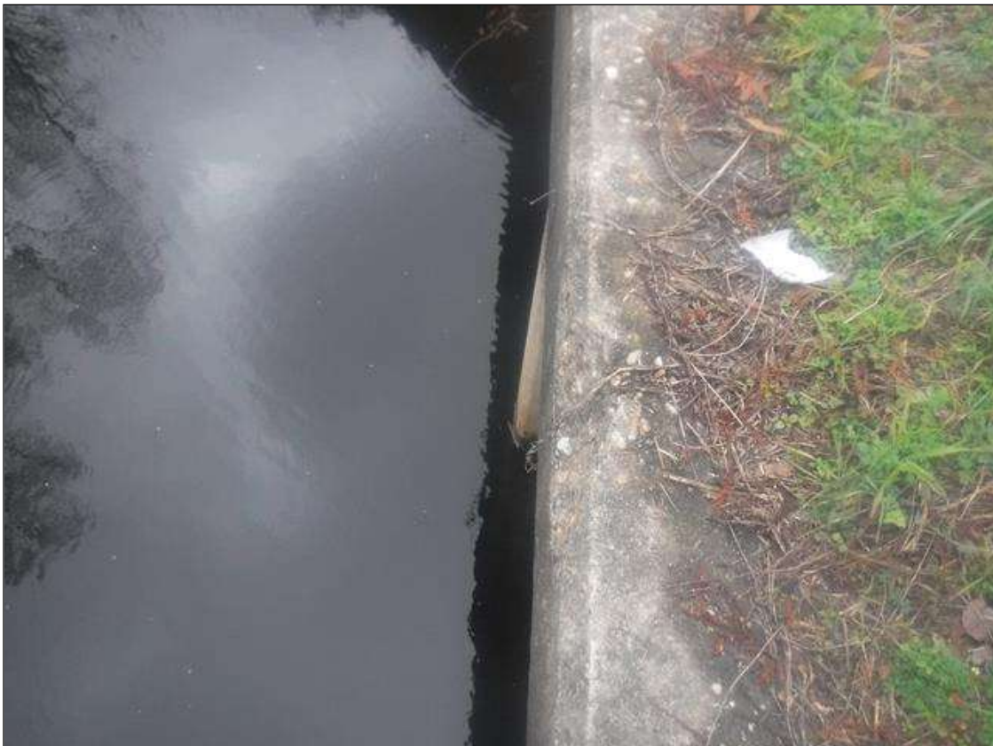
SPALL ON WEST HEADWALL, OVER BARREL 1
