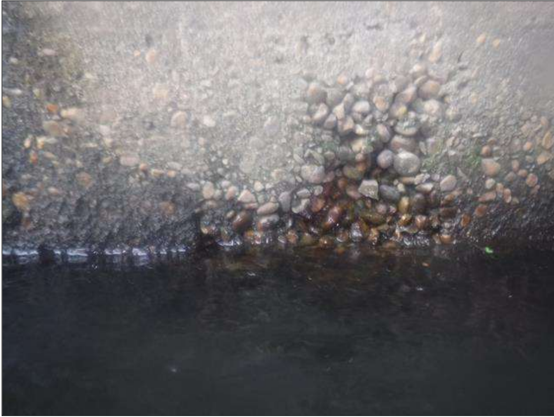
Span 1 Culvert Section 1: VOID ON THE EXTERIOR WALL. 8" DIAMETER X 2" DEEP. 1' FROM THE EAST END/ 5.5' ABOVE BOTTOM SLAB
