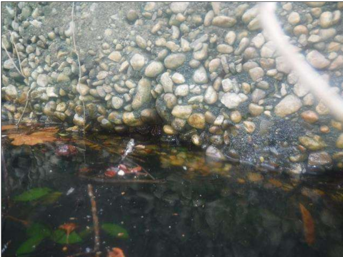
VOID ON THE SE WINGWALL. 3"V X 1"W X 2"DEEP
