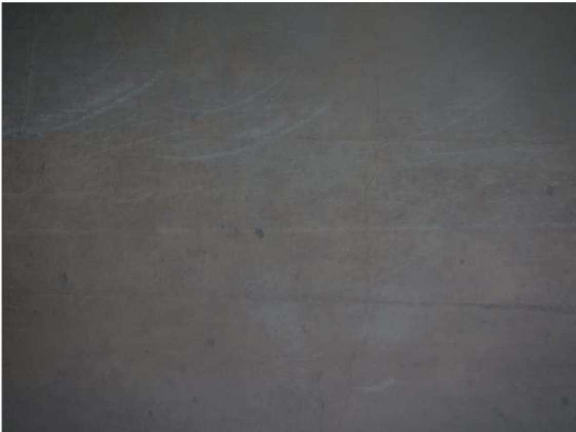
Span 2 Culvert Section 1: H/L VERTICAL CRACKING ON INTERIOR WALL NEAR C/L
