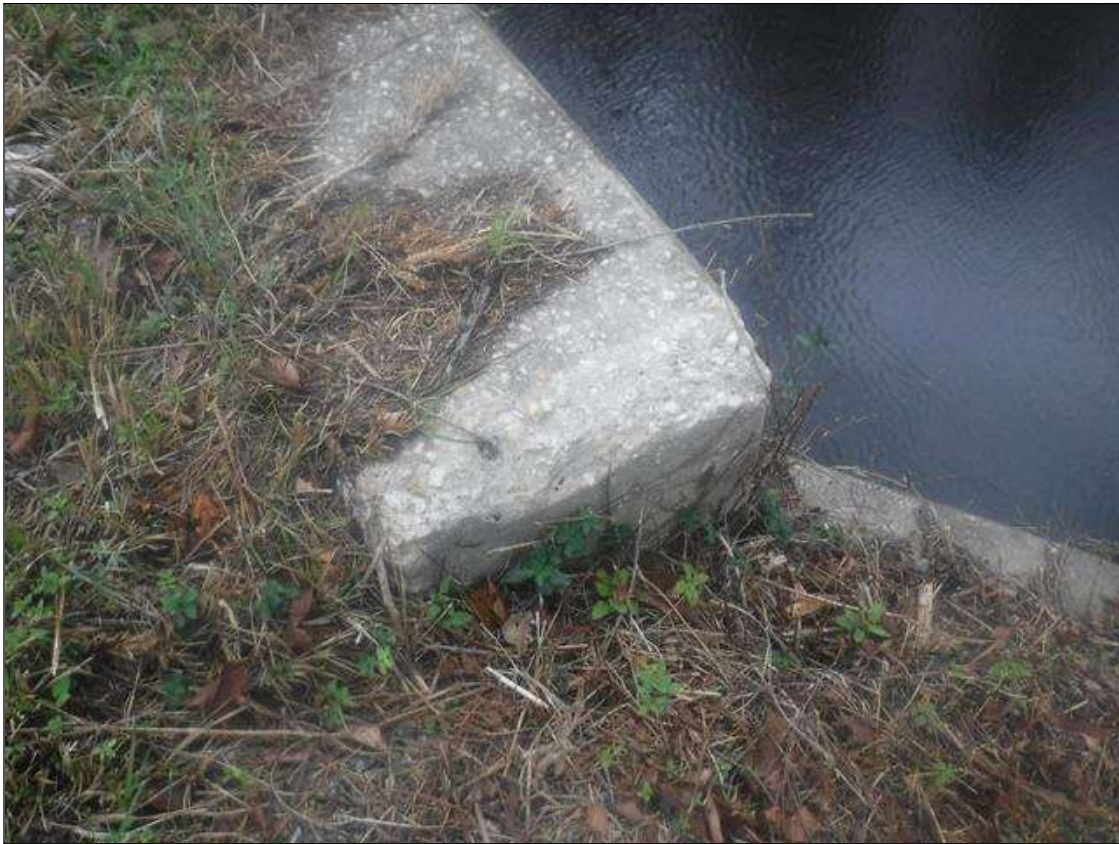
SPALL ON EAST HEADWALL, SOUTH END
