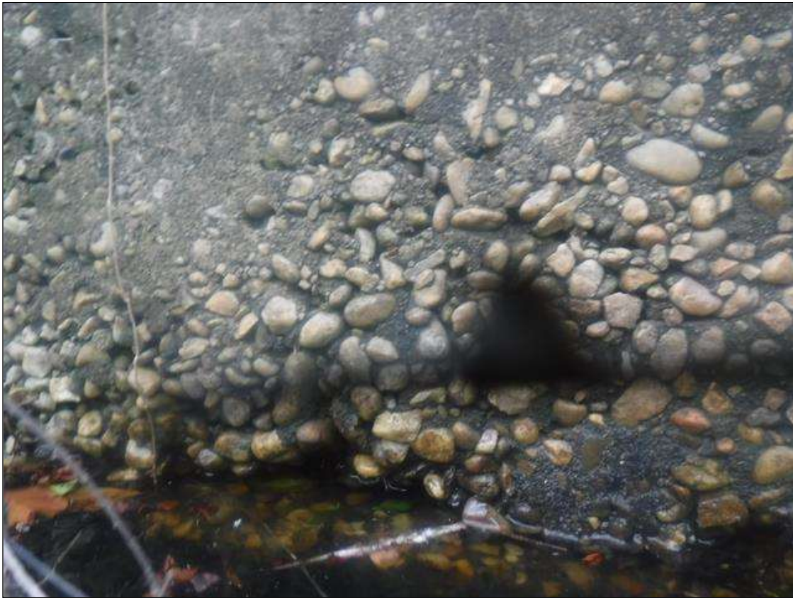
COARSE AGGREGATE EXPOSED ON WING (ALL WINGS SIMILIAR)
