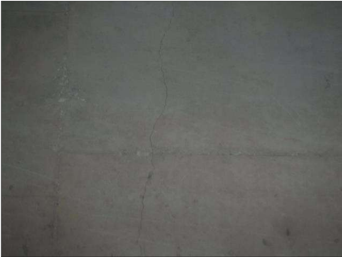
Span 1 Culvert Section 1: H/L VERTICAL CRACK ON INTERIOR WALL NEAR C/L
