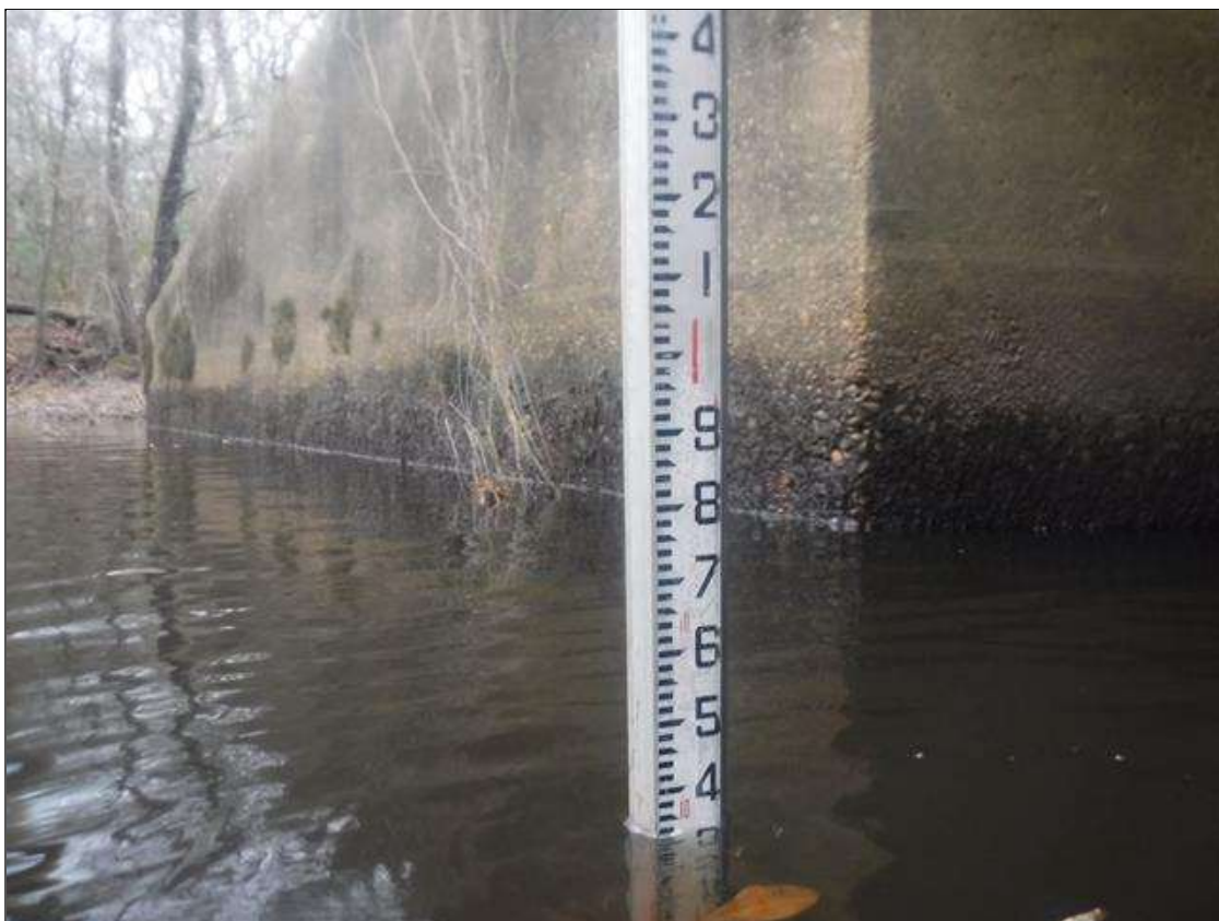
Span 3 Culvert Section 1: UPSTREAM CURTAIN WALL EXPOSURE 3.0' VERT. WITH 0.5' VERT. BELOW CURTAINWALL X 0.5' PROBE. (PAR)
