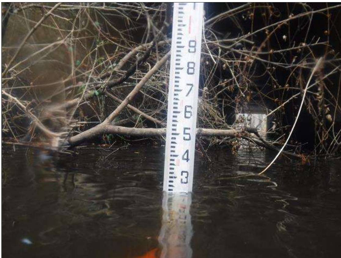
Span 2 Culvert Section 1: UPSTREAM CURTAIN WALL EXPOSURE 2.7' WITH 0.5' VERT. BELOW CURTAINWALL WITH PROBE TO 0.5'. DOWNSTREAM CURTAIN WALL EXPOSURE 1.1' VERT. (PAR)
