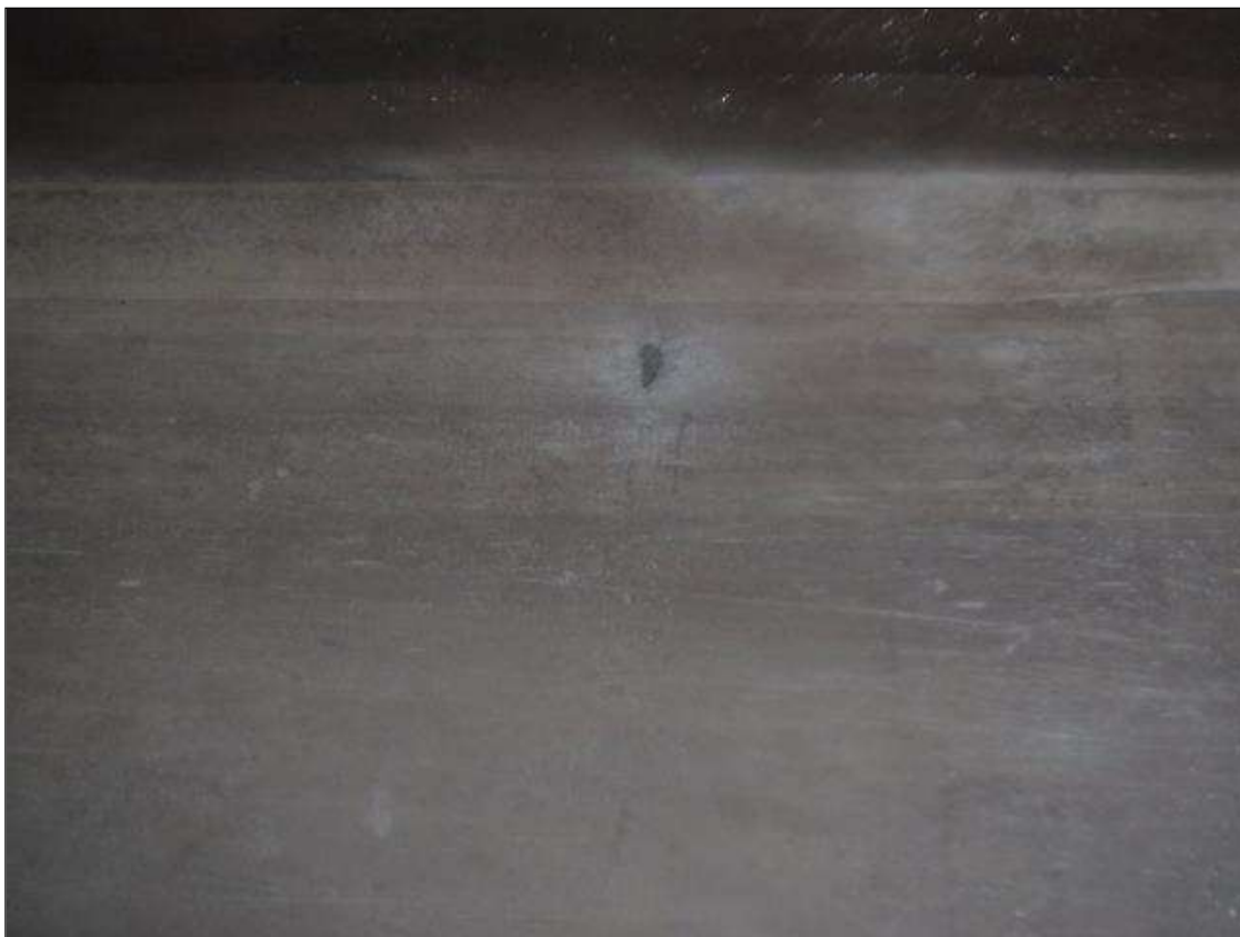
Span 2 Culvert Section 1: REBAR EXPOSED, SECTION LOSS DUE TO SPALLS ON INTERIOR WALL 2, 15' FROM EAST END. (PAR)
