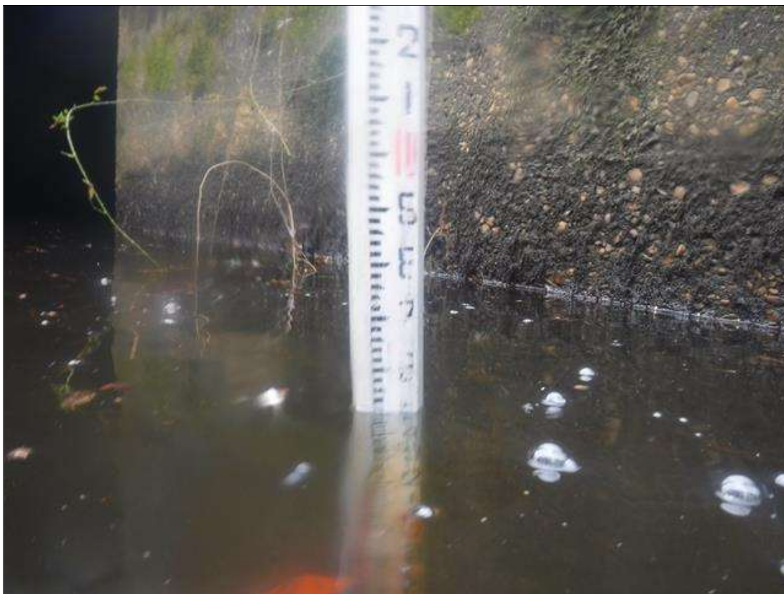
SCOUR AT SW WING (PAR)
