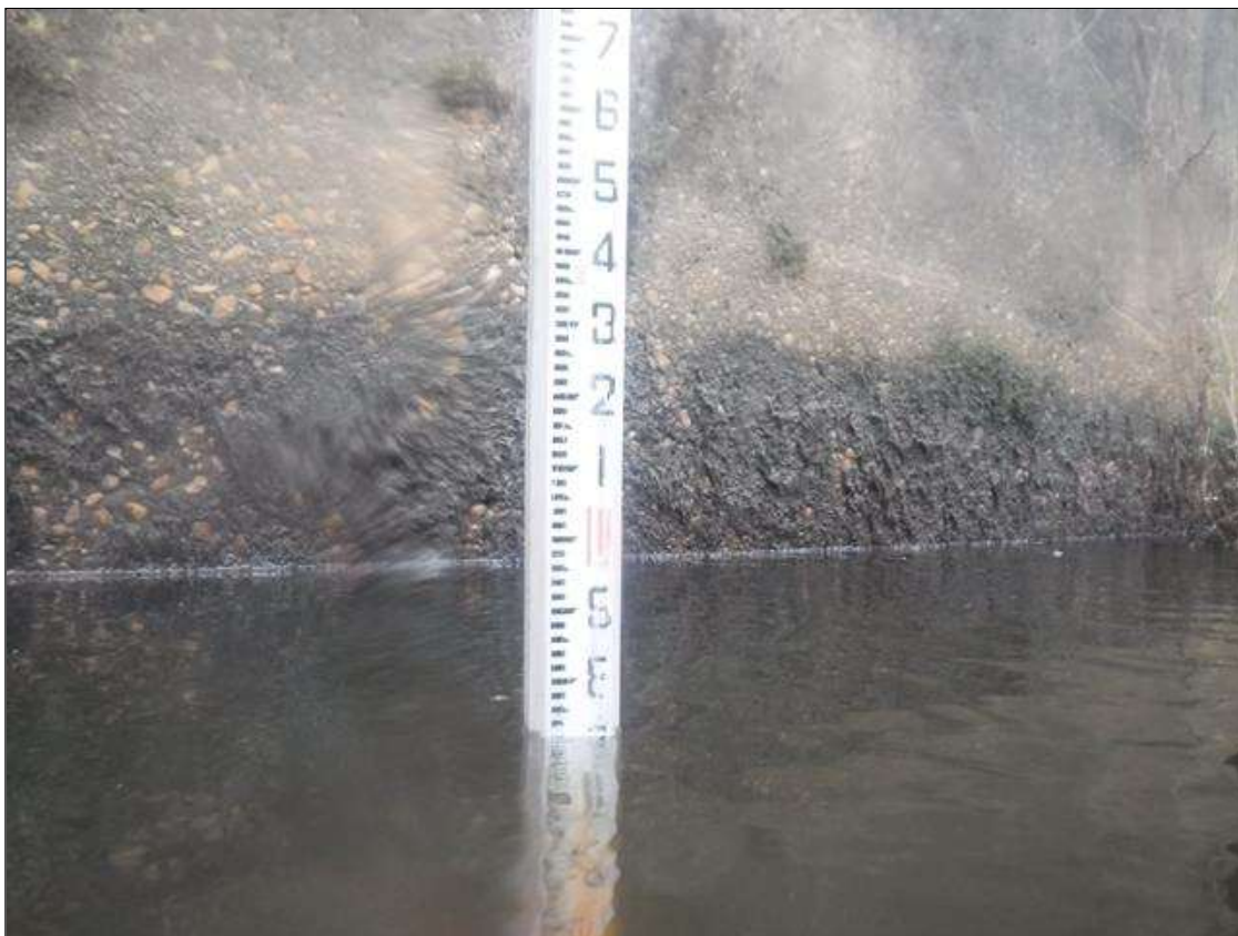
NW WING SCOUR (PAR)
