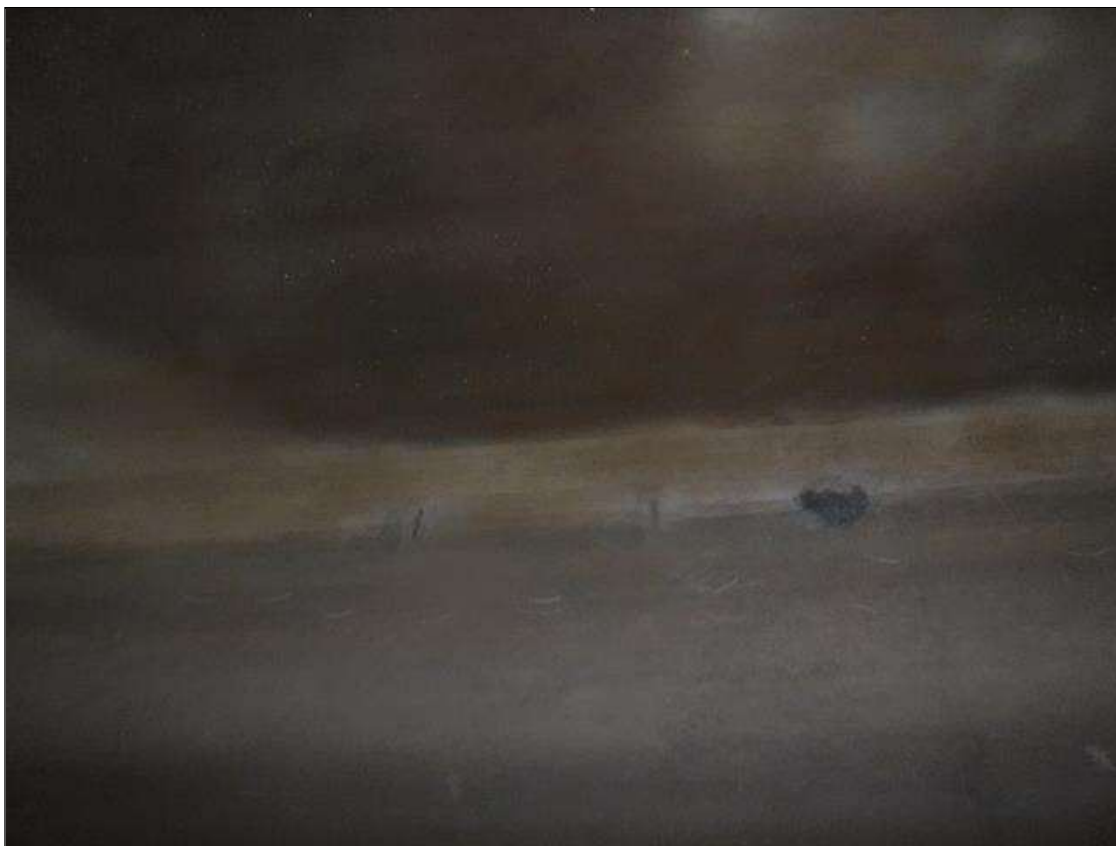
Span 2 Culvert Section 1: TOP SLAB SPALLS NEAR C/L- 9' LONG X 8" WIDE X 1" DEEP. SPALL ON INTERIOR WALL 1, 20' FROM WEST END.
