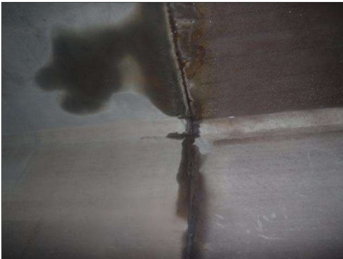
Span 1 Culvert Section 1: CONSTRUCTION JOINTS OPEN TO 1/16" WITH EFFLORESCENCE/WATER LEAKAGE (ALL BARRELS SIMILIAR)
