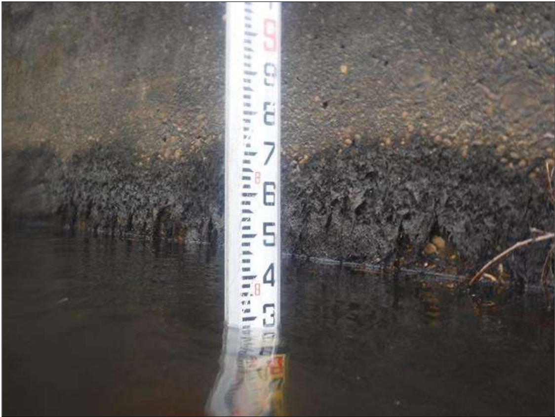
NE WING, SCOUR (PAR)
