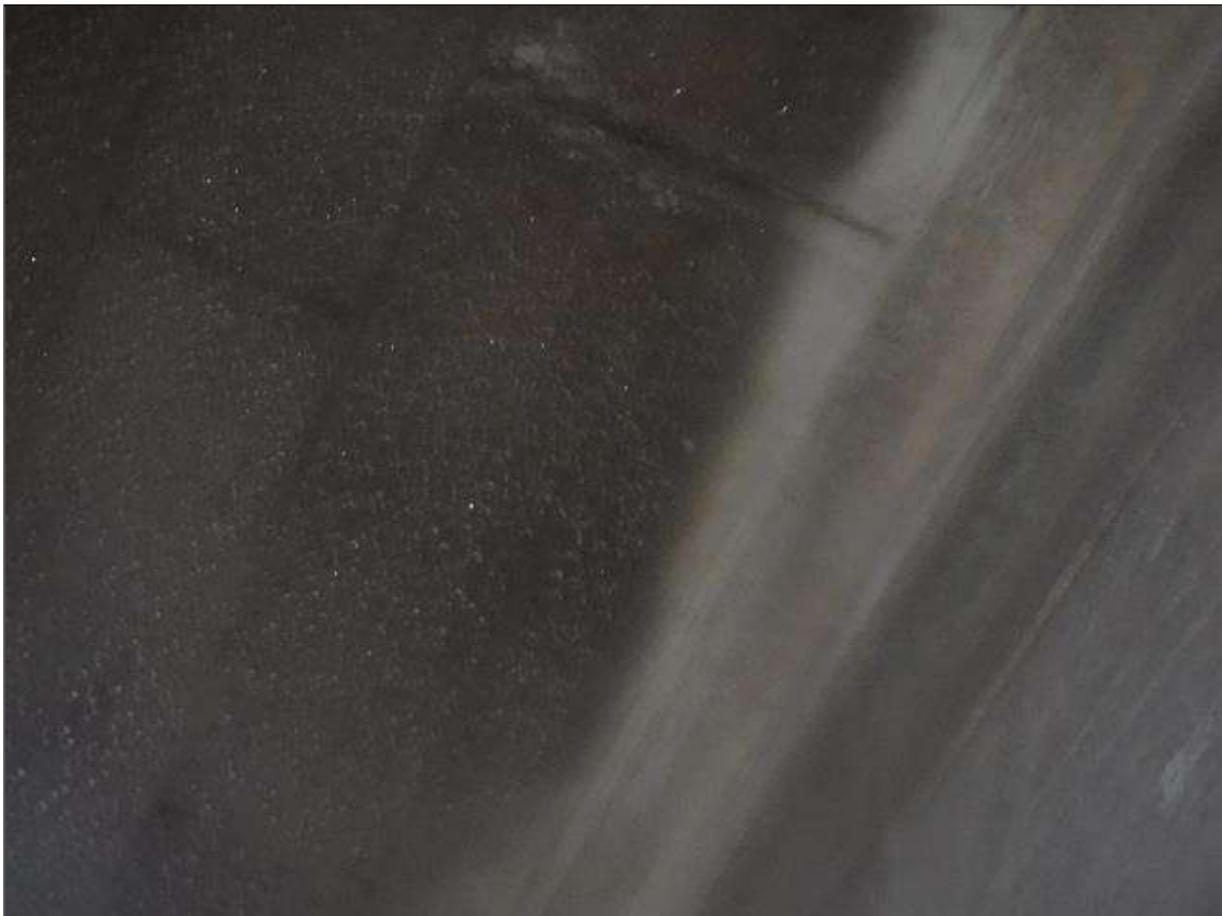
Span 2 Culvert Section 1: TOP SLAB SPALLS NEAR C/L- 9' LONG X 8" WIDE X 1" DEEP. SPALL ON INTERIOR WALL 1, 20' FROM WEST END.
