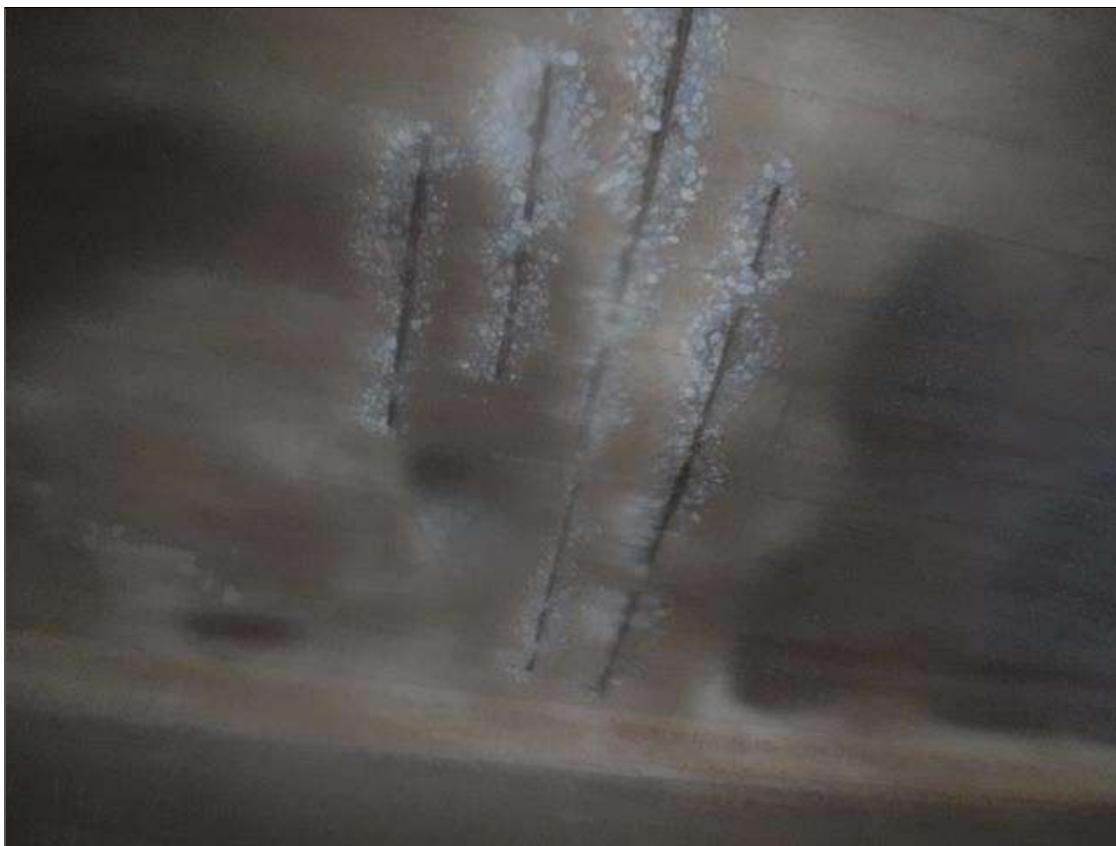
Span 1 Culvert Section 1: 5 AREAS OF SPALLS- 6' LONG X 8" WIDE X 1" DEEP (PAR)
