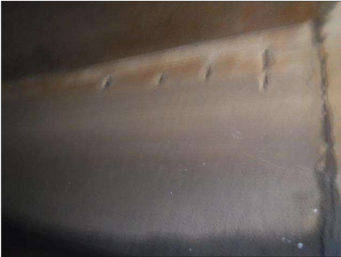
Span 2 Culvert Section 1: TOP SLAB SPALLS NEAR C/L- 9' LONG X 8" WIDE X 1" DEEP. SPALL ON INTERIOR WALL 1, 20' FROM WEST END.
