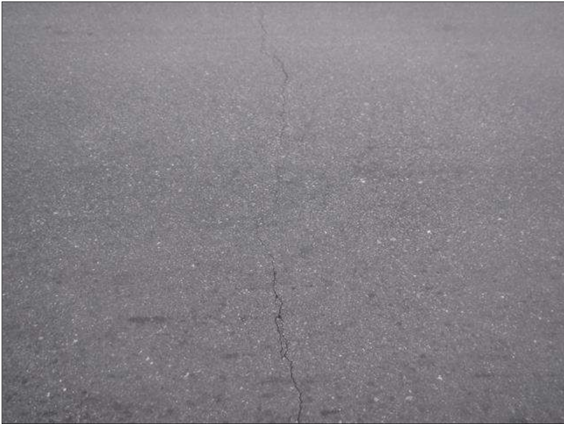
CRACKING IN AWS UP TO 1/8"
