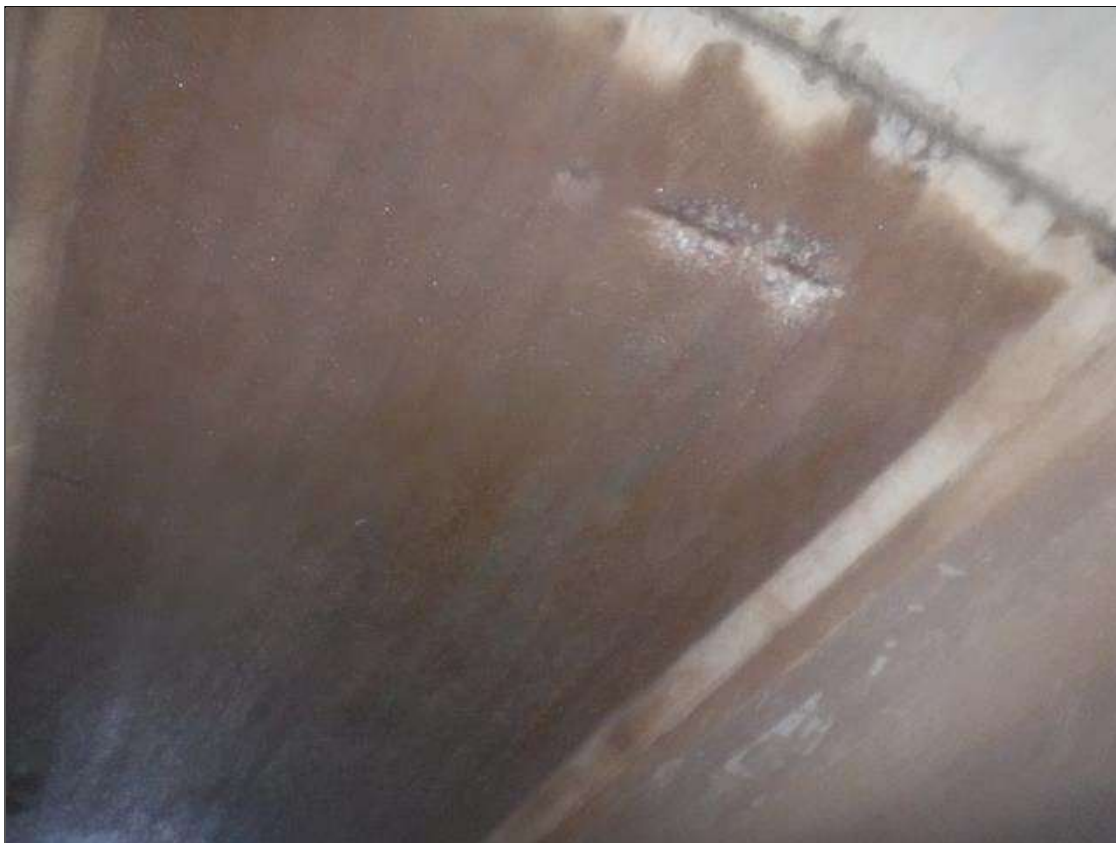
Span 3 Culvert Section 1: REBAR EXPOSED, SECTION LOSS DUE TO SPALLS ON TOP SLAB. (PAR)
