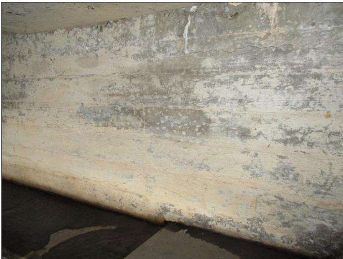
End Bent 2 Abutment: MULTIPLE HORZ. CRACKS UP TO 1/16TH IN WIDE THRU OUT END BENT BACKWALL AT OUTSIDE FACES.
