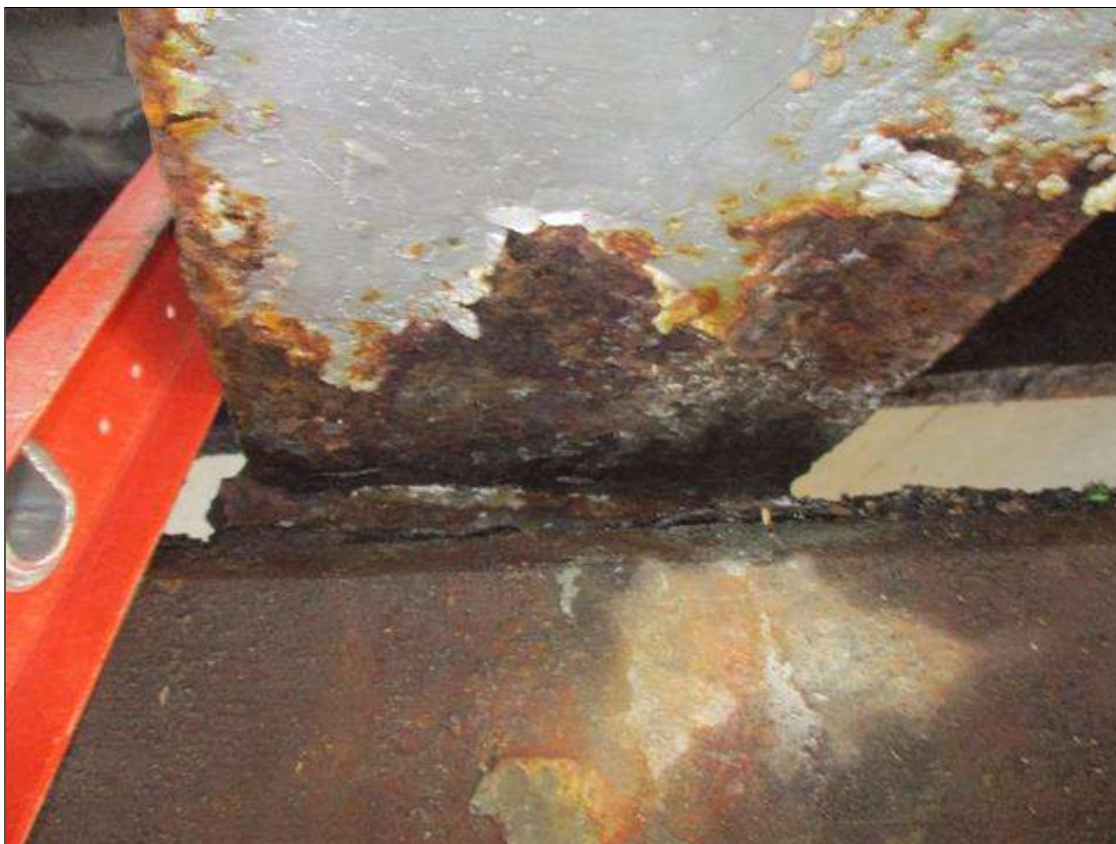
Span 2 Beam 4: BTM FLANGE SECTION LOSS (27% SL, 1/4IN SL, 11/16IN REMAIN) FULL WIDTH FOR 16IN FAR END. (PAR)
