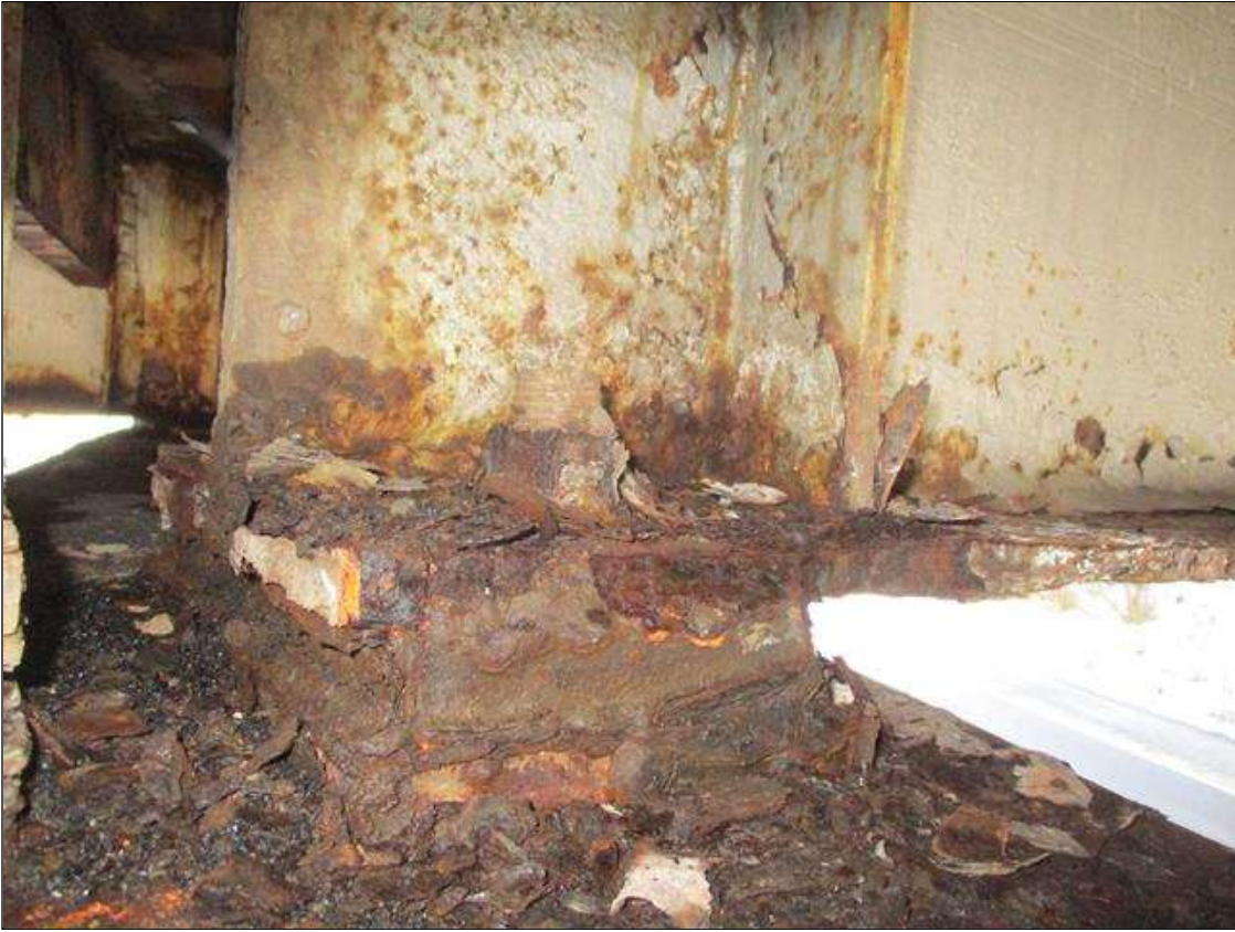
Span 3 Beam 5: BTM FLANGE SECTION LOSS (40% SL, 3/8IN SL, 9/16IN REMAIN) FULL WIDTH FOR 1FT AT NEAR END. (PAR)
