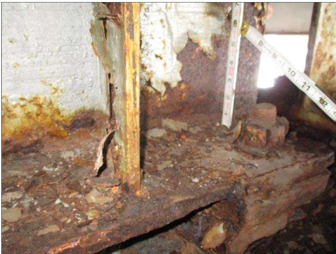
Span 4 Beam 6: WEB SECTION LOSS NEAR TOP AND BOTTOM FLANGE, 1/2IN REMAIN X 1.5 FT HIGH FOR 6 IN LONG
