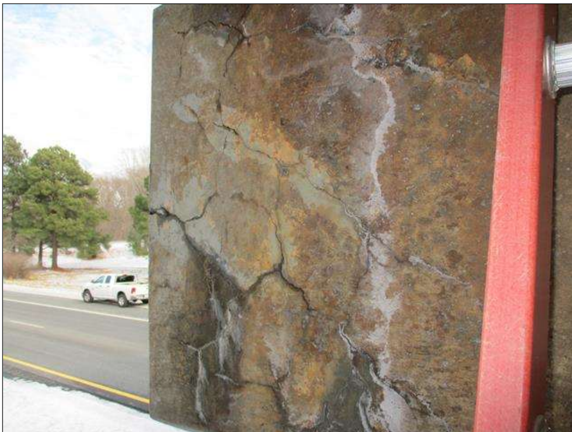
Bent 2 Cap 1: HORZ. & MAP CRACKING (UP TO 1/8IN) WEST/ EFFLO. & RUSTING STAINING THRU OUT ALL FACES OF CAP
