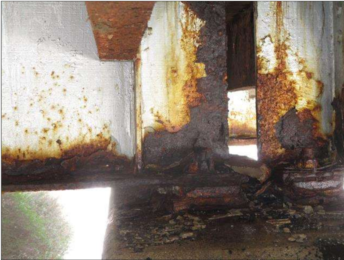
Span 1 Beam 9: BTM FLANGE SECTION LOSS (40% SL, 3/8IN SL, 9/16IN REMAIN) FULL WIDTH FOR 2FT AT FAR END. STIFFENER SECTION LOSS (1/4IN REMAIN) 3IN HIGH X 3IN WIDE TO LEFT SIDE STIFFENER AT FAR END (PAR)
