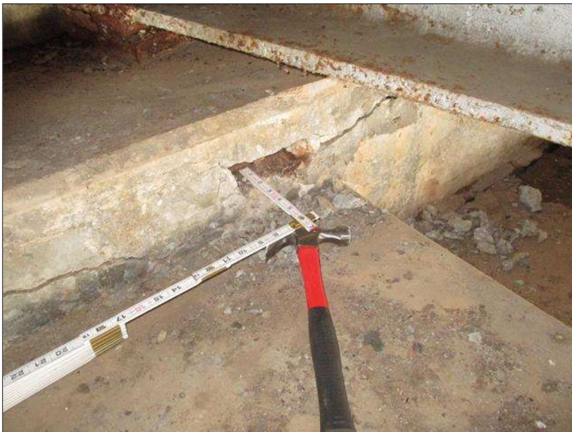
End Bent 2 Cap 1: SPALL WITH EXPOSED REBAR UP TO 9 IN LONG X 5" HIGH X 2.5" DEEP UNDER GIRDER 8. EXPOSED REBAR HAS NO SECTION LOSS
