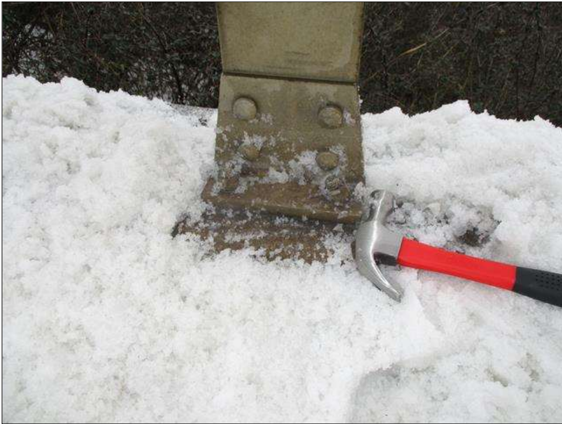
Span 1 Left Bridge Rail: MINOR DAMAGE & BENT ANCHOR AT 3RD POST (POST REMAINS SECURE)
