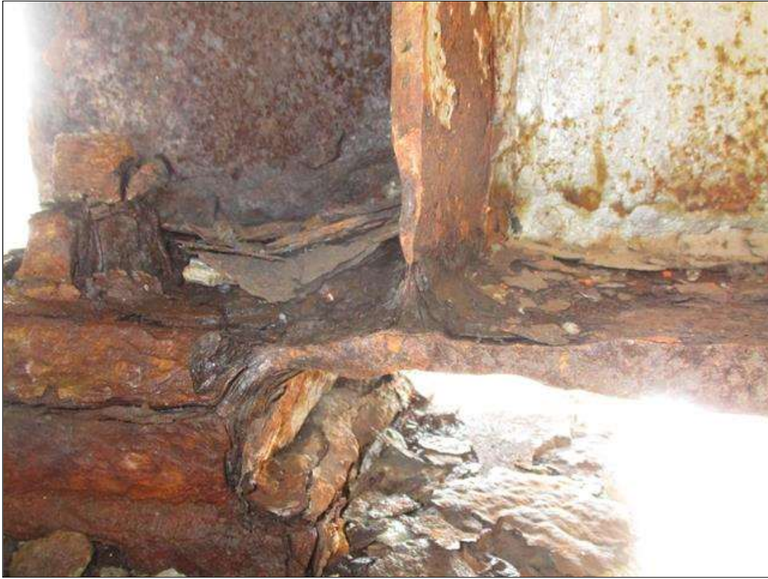
Span 1 Beam 10: WEB SECTION LOSS (3/16IN SL, 7/16 REMAIN) X FULL HEIGHT FOR 8IN AT FAR END. STIFFENER SECTION LOSS (1/4IN REMAIN) 2IN HIGH X 3IN WIDE TO LEFT SIDE STIFFENER AT FAR END. (PAR)
