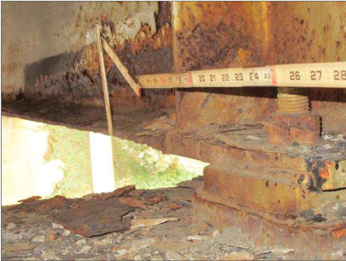
Span 3 Beam 7: BTM FLANGE SECTION LOSS (60% SL, 9/16IN SL, 3/8IN REMAIN) FULL WIDTH & WEB PITTING (1/2IN REMAIN) X 6IN HIGH FOR 5FT AT NEAR END. (PAR)
