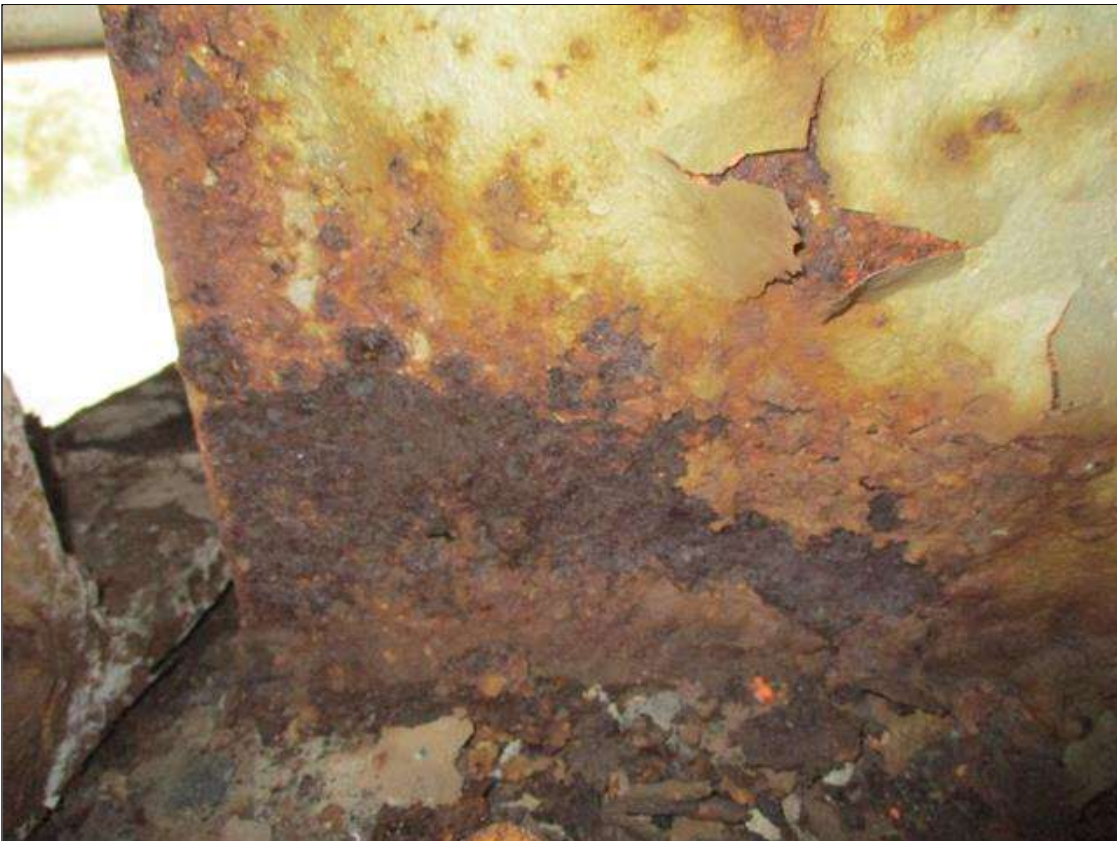
Span 2 Beam 3: WEB SECTION LOSS UP TO 100% FOR A 1 IN DIAMETER AT NEAR BOTTOM OF WEB. AVERAGE 3/8IN REMAINING X 4IN HIGH FOR 8IN AT FAR END. (PAR)
