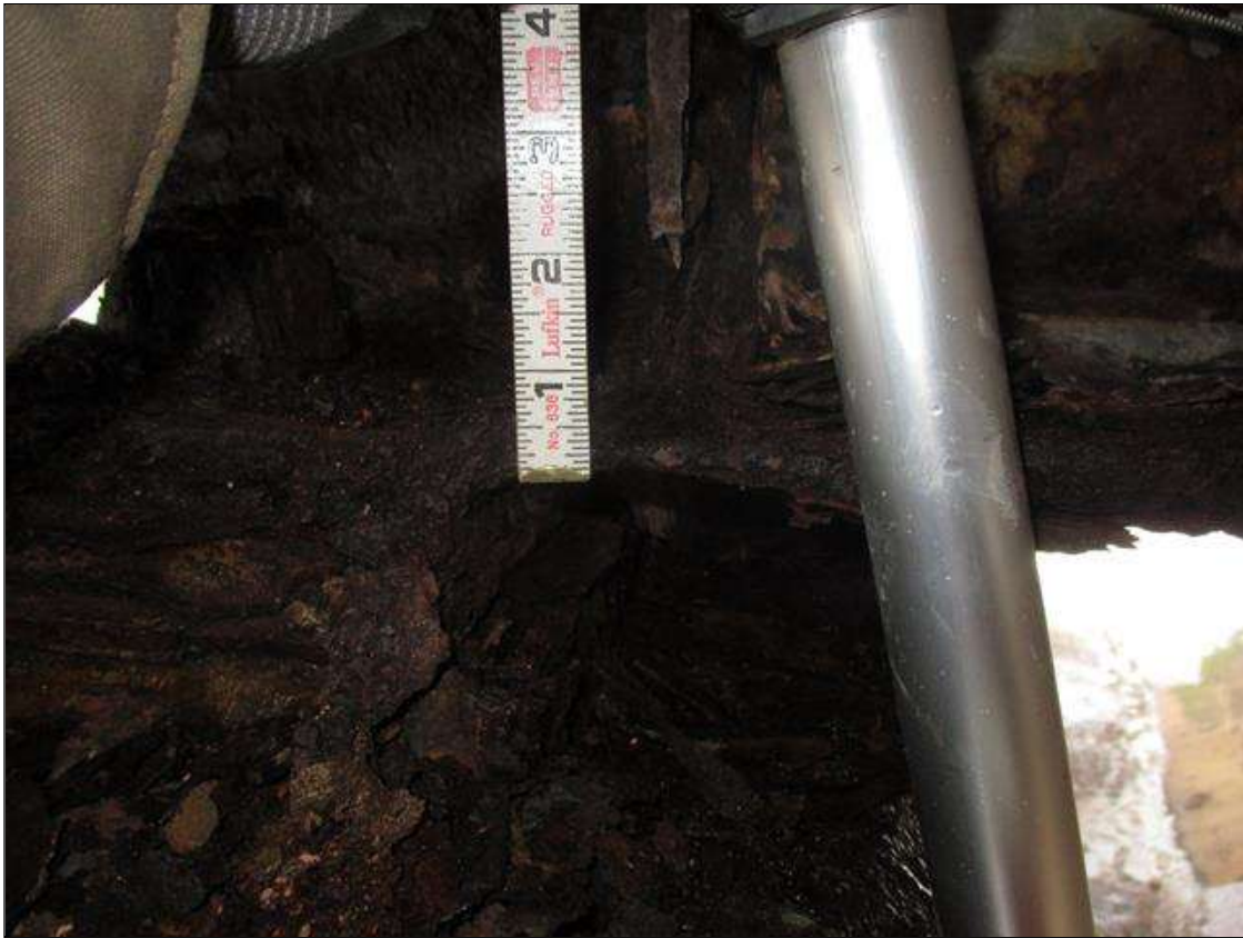
Span 4 Beam 8: BTM FLANGE SECTION LOSS, 7/16IN REMAINING, FULL WIDTH FOR 2FT AT NEAR END. (PAR)
