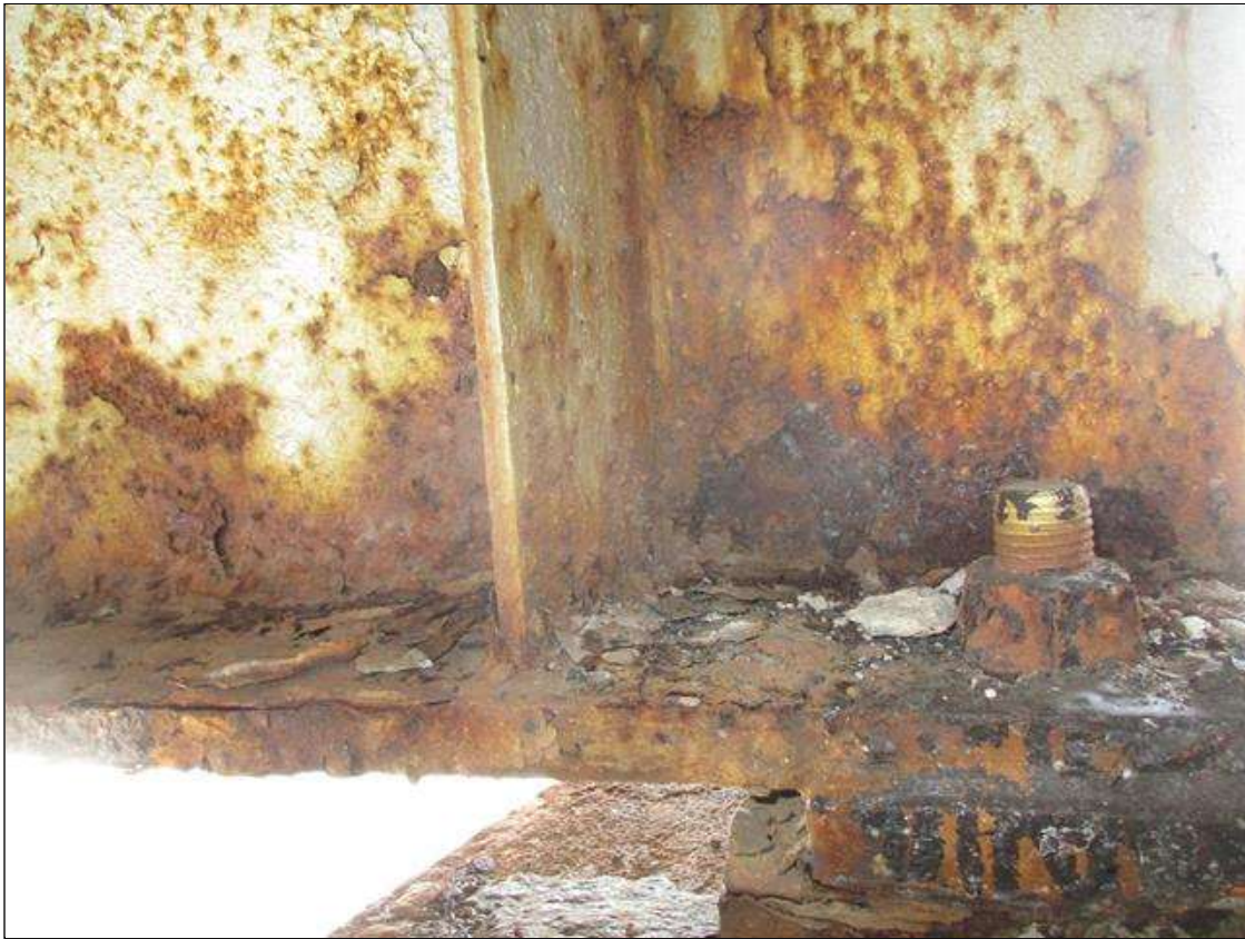
Span 2 Beam 10: NO SIGNIFICANT SECTION LOSS IN THE BTM FLANGE. SECTION LOSS IN THE WEB WITH PITTING (1/2IN REMAIN) X 6IN HIGH FOR 8FT AT NEAR END. (PAR)
