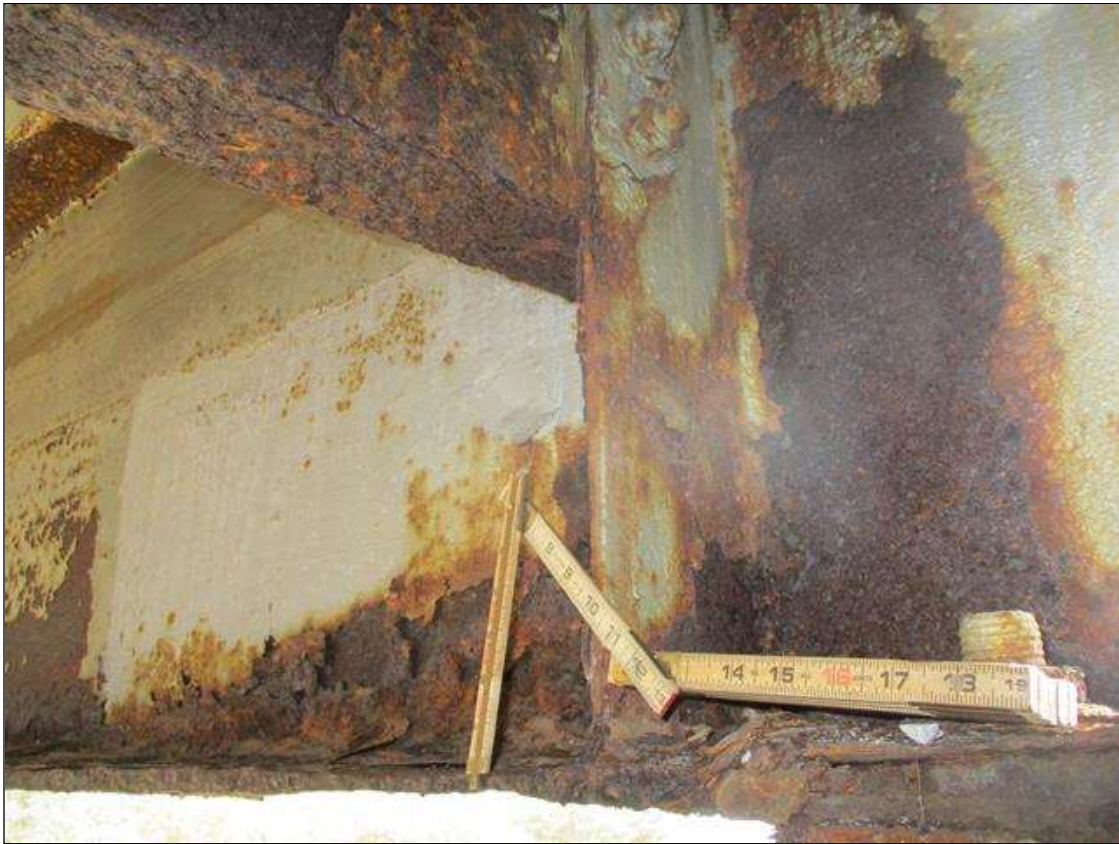
Span 3 Beam 10: BTM FLANGE SECTION LOSS (40% SL, 3/8IN SL, 9/16IN REMAIN) FULL WIDTH & WEB PITTING (1/8IN REMAIN) X FULL HEIGHT FOR 6 INCHES AT NEAR END. (PAR)
