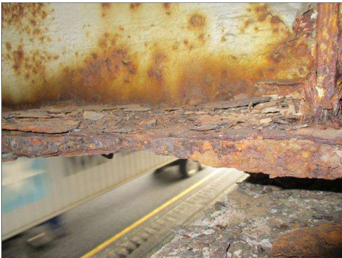
Span 3 Beam 3: BTM FLANGE SECTION LOSS (53% SL, 1/2IN SL, 7/16IN REMAIN) FULL WIDTH FOR UP TO 3FT AT NEAR END. (PAR)
