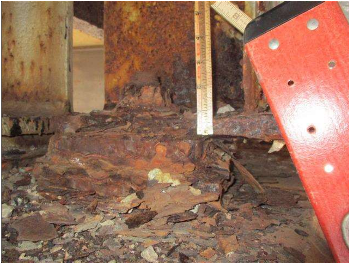
Span 2 Beam 7: BTM FLANGE SECTION LOSS (33% SL, 5/16IN SL, 5/8IN REMAIN) FULL WIDTH FOR 4IN AT FAR END. (PAR)
