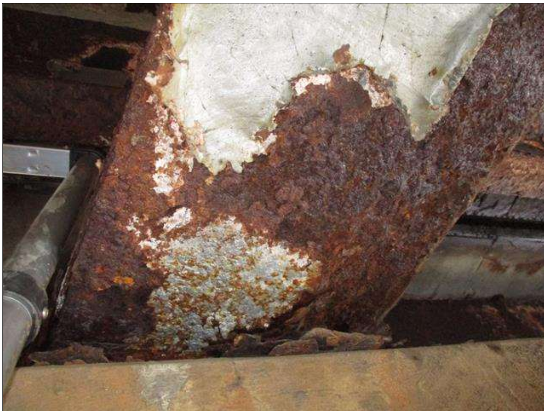
Span 4 Beam 3: BTM FLANGE SECTION LOSS (62% SL, 1/2IN SL, 5/16IN REMAIN) 4 IN WIDE FOR 1FT AT NEAR END. (PAR)
