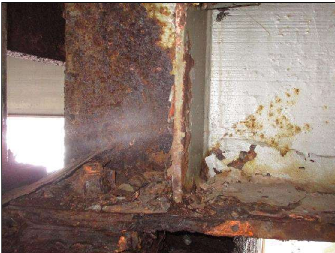
Span 4 Beam 7: BTM FLANGE SECTION LOSS (62% SL, 1/2IN SL, 5/16IN REMAIN) FULL WIDTH & WEB PITTING (9/16IN REMAIN) X 4IN HIGH FOR 2.5FT AT NEAR END.(PAR)
