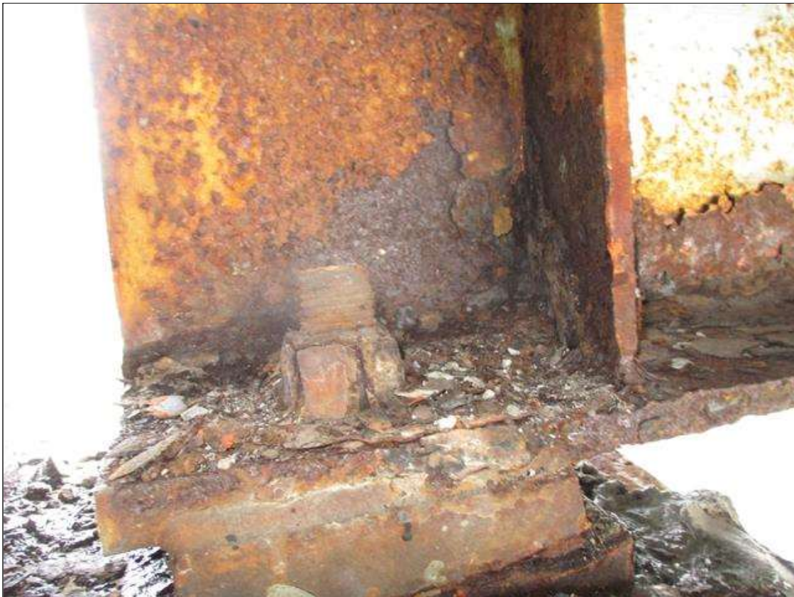
Span 2 Beam 1: BTM FLANGE SECTION LOSS (40% SL, 3/8IN SL, 9/16IN REMAIN) FULL WIDTH & WEB PITTING (9/16IN REMAIN) X 4IN HIGH FOR 4FT AT NEAR END. (PAR)
