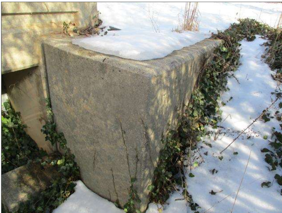
SOME MINOR EFFLOR AT SOUTHEAST WINGWALL, TYPICAL
