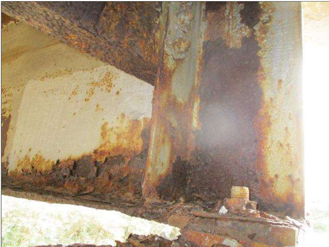
Span 3 Beam 10: BTM FLANGE SECTION LOSS (40% SL, 3/8IN SL, 9/16IN REMAIN) FULL WIDTH & WEB PITTING (1/8IN REMAIN) X FULL HEIGHT FOR 6 INCHES AT NEAR END. (PAR)
