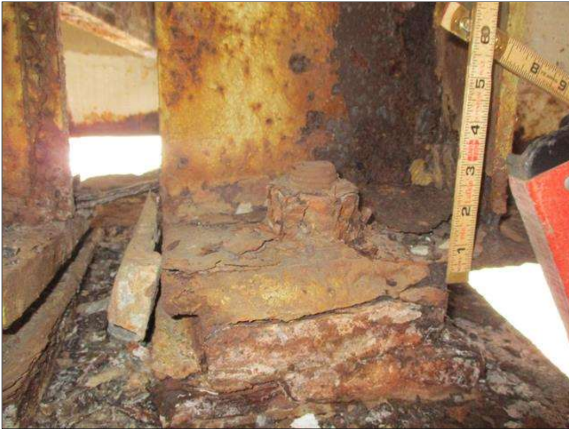
Span 2 Beam 9: BTM FLANGE SECTION LOSS (66% SL, 5/8IN SL, 5/16IN REMAIN) FULL WIDTH & WEB PITTING (9/16IN REMAIN) X 3IN HIGH FOR 2FT AT FAR END. (PAR)
