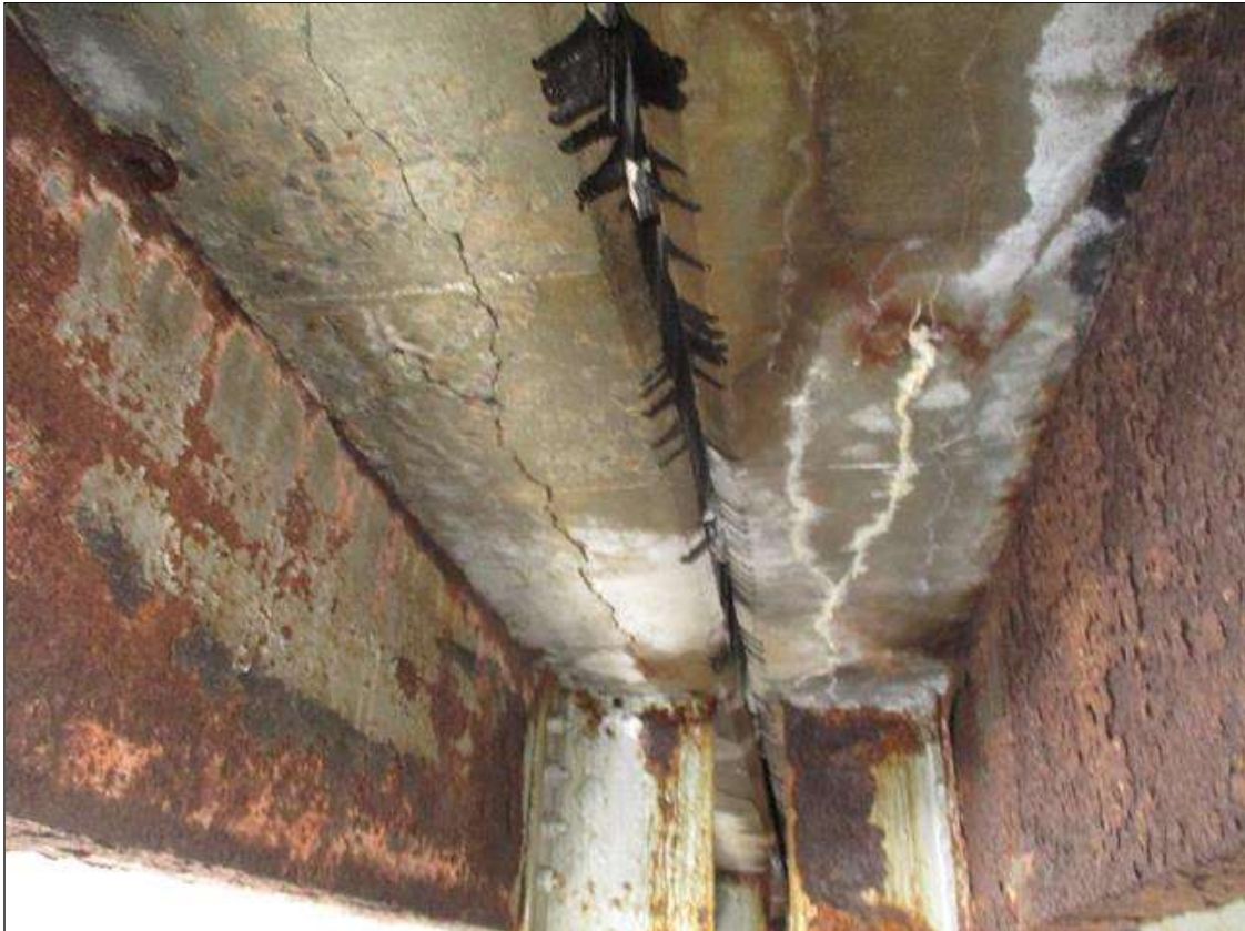
Span 4 Deck: TRANSVERSE CRACKING UP TO 1/4 IN WIDE FOR FULL WIDTH IN BAY 8 AND 9 WITH DELAMINATED AREA SURROUNDING THE CRACK UP TO 4 IN WIDE
