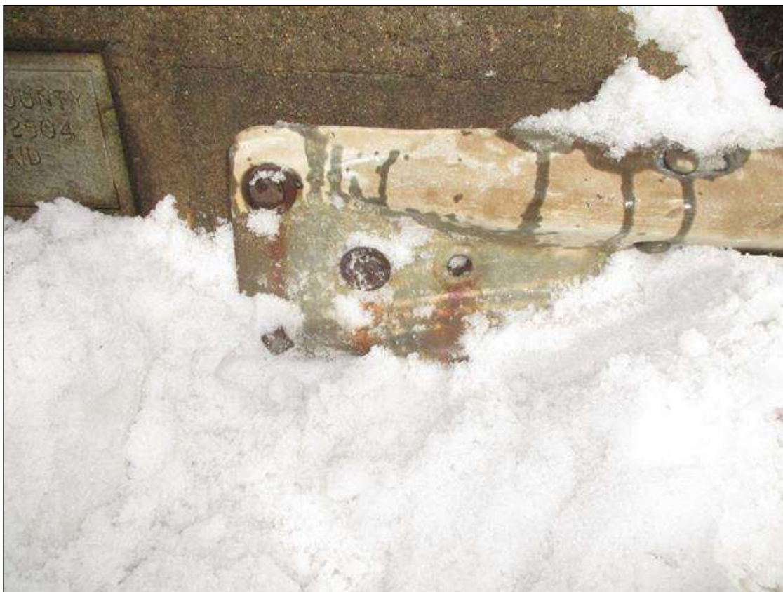
Span 4 Left Bridge Rail: 1X MISSING BOLT & 1IN SEPERATION OF GUARDRAIL ATTACHMENT AT FAR END (ATTACHMENT REMAINS SECURE)
