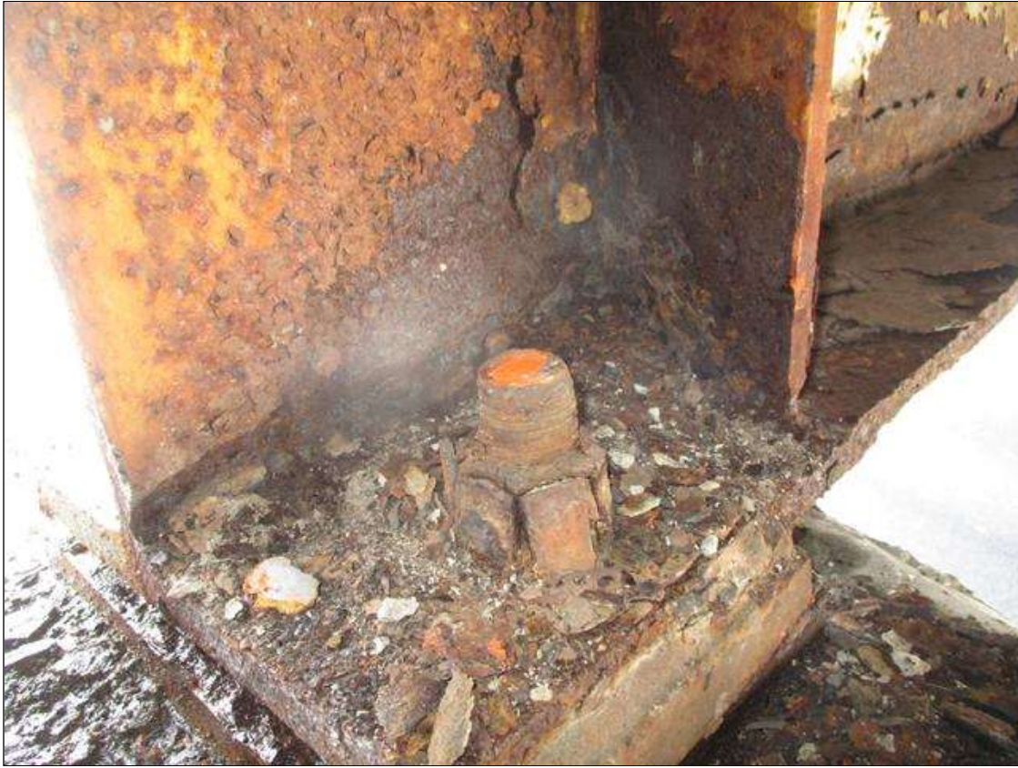
Span 2 Beam 1: BTM FLANGE SECTION LOSS (40% SL, 3/8IN SL, 9/16IN REMAIN) FULL WIDTH & WEB PITTING (9/16IN REMAIN) X 4IN HIGH FOR 4FT AT NEAR END. (PAR)
