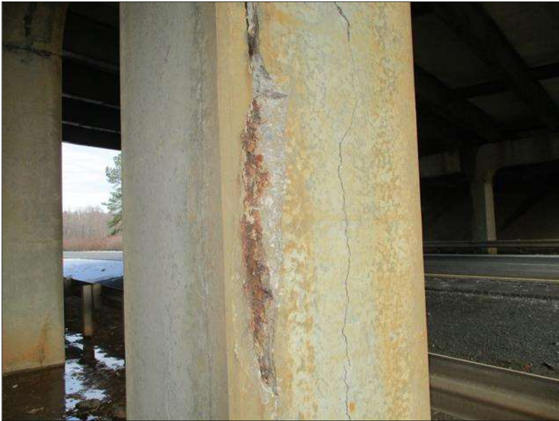
Bent 2 Pile 4: SPALL WITH EXPOSED REBAR IN THE SOUTH FACE OF COLUMN UP TO 4 FT HIGH X 5 IN WIDE X 2.5 IN DEEP STARTING 3 FT FROM GROUND LINE. UP TO 80% SECTION REMAINING ON THE EXPOSED REBAR. COLUMN IS DELAMINATED ABOVE THE SPALL FOR THE REMAINDER OF THE COLUMN HEIGHT
