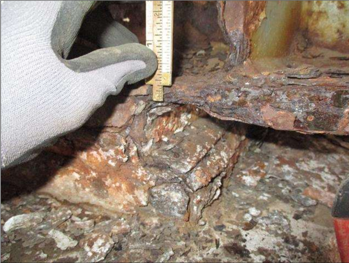
Span 2 Beam 3: BTM FLANGE SECTION LOSS (35% SL, 1/2IN SL, 7/16IN REMAIN) 4IN WIDE AT BOTH SIDES FOR 6IN AT FAR END. (PAR)
