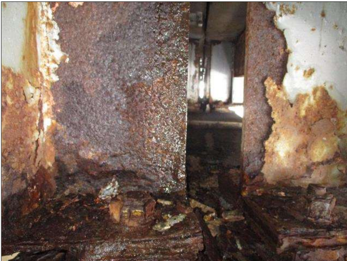
Span 4 Beam 4: WEB SECTION LOSS (3/16IN SL, 7/16IN REMAIN) X UP TO FULL HEIGHT FOR 10IN AT NEAR END. (PAR)
