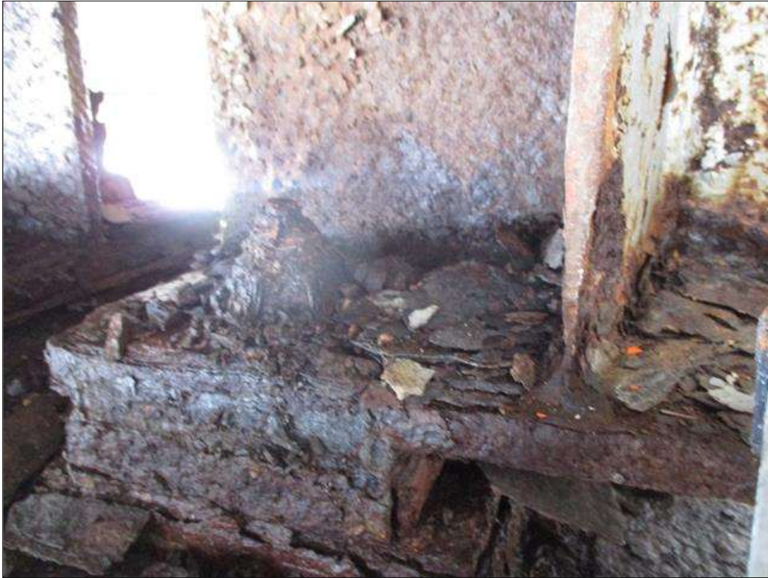
Span 1 Beam 2: BTM FLANGE SECTION LOSS (33% SL, 5/16IN SL, 5/8IN REMAIN) FULL WIDTH & WEB PITTING (9/16IN REMAIN) X 3IN HIGH FOR 2FT AT FAR END. STIFFENER SECTION LOSS (1/4IN REMAIN) 3IN HIGH X 2IN WIDE TO LEFT SIDE STIFFENER AT FAR END. (PAR)
