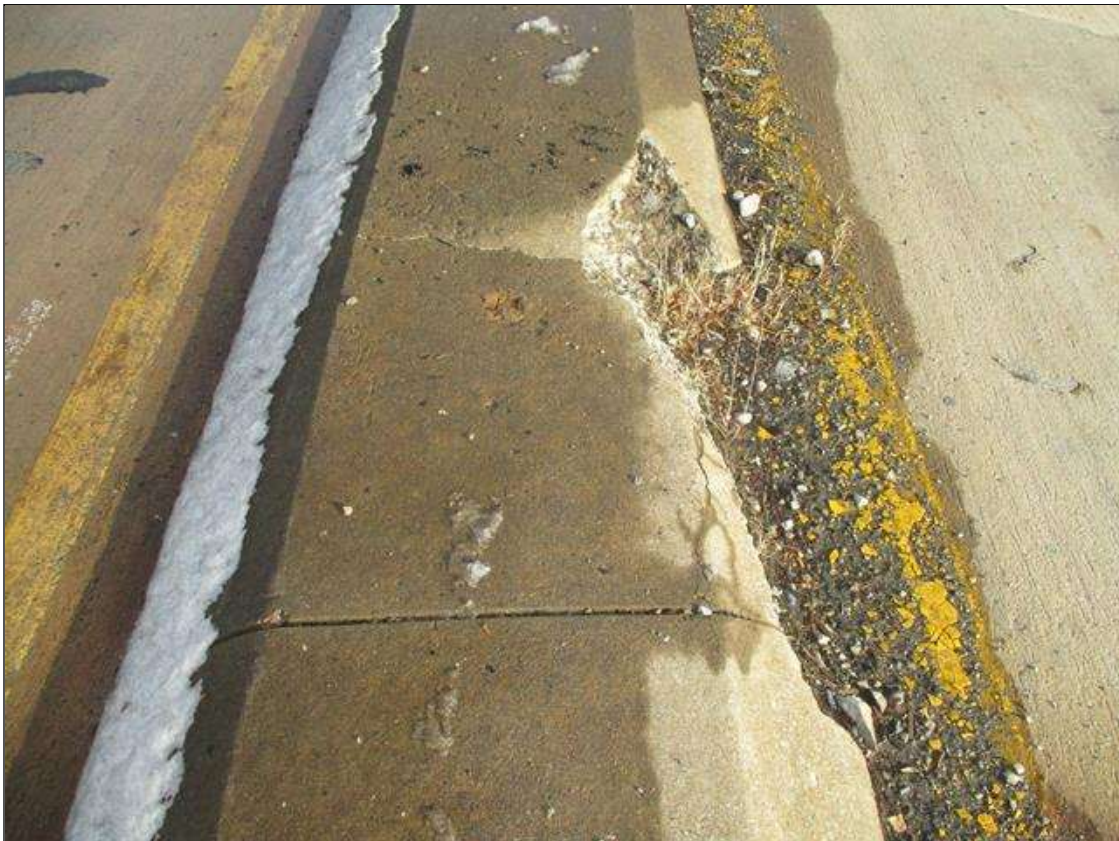
Span 4 Deck: SPALL(6FT X 12IN X 6IN DEEP) TO RIGHT SIDE OF MEDIAN, 15FT FROM FAR END. SPALL (15FT X 4IN X 4IN) TP LEFT EDGE OF MEDIAN AT FAR END.
