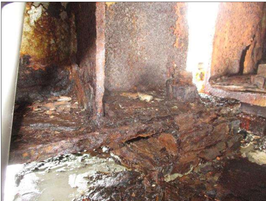
Span 1 Beam 1: BTM FLANGE SECTION LOSS (47% SL, 7/16IN SL, 1/2IN REMAIN) FULL WIDTH & WEB PITTING (9/16IN REMAIN) X 3IN HIGH FOR 3FT AT FAR END. (PAR)
