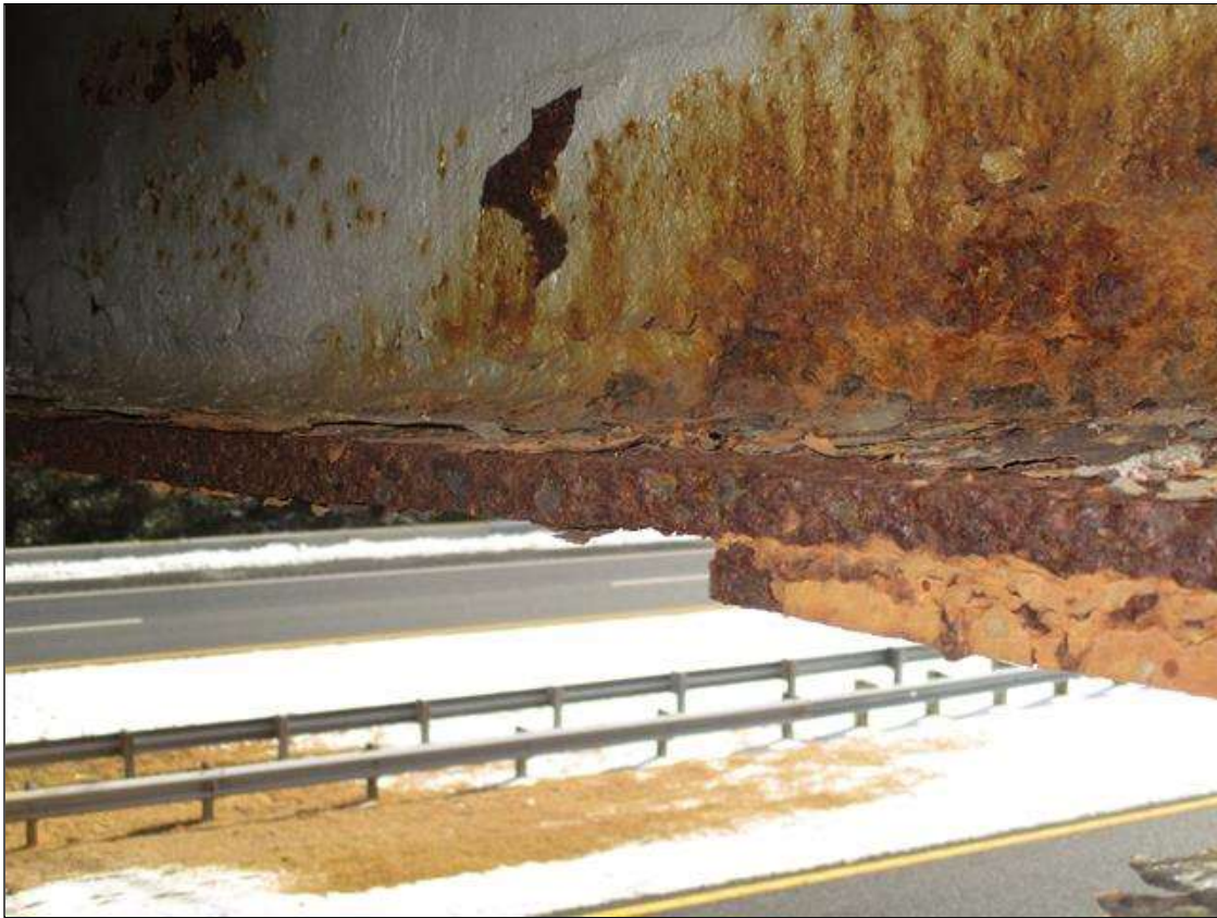
Span 2 Beam 8: BTM FLANGE SECTION LOSS (27% SL, 1/4IN SL, 11/16IN REMAIN) FULL WIDTH FOR 1FT STARTING AT 1FT FROM NEAR END AFTER REPAIR PLATE. (PAR)
