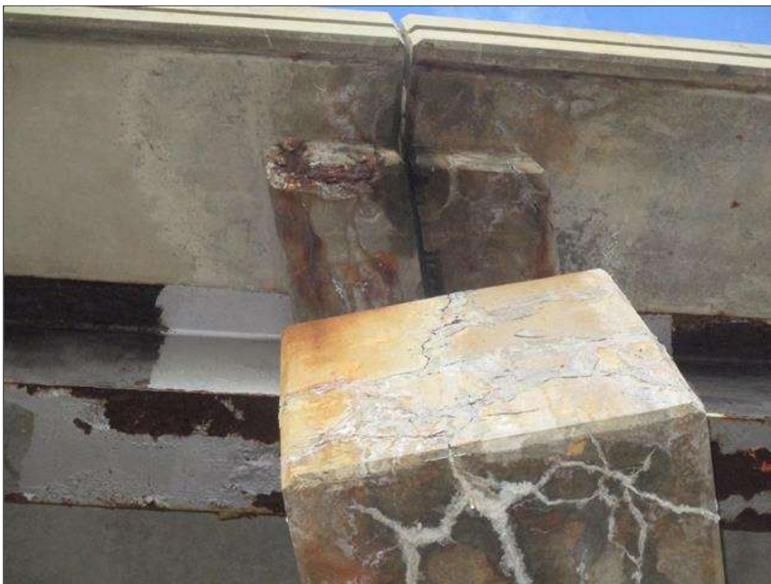
Span 2 Deck: SPALL (1FT X 8IN X 2IN) WEST/ EXPOSED REBAR TO RIGHT SIDE OVERHANG HAUNCH OVER BENT 2. UP TO 90% SECTION REMAINING IN THE EXPOSED REBAR. (PAR)
