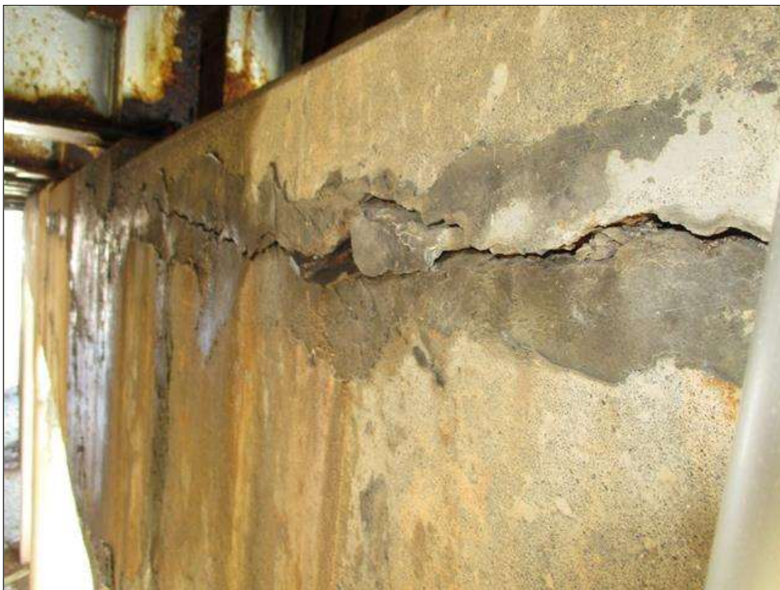
Bent 1 Cap 1: HORZ. & MAP CRACKING (UP TO 1/8IN) WEST/ EFFLO. & RUSTING STAINING THRU OUT ALL FACES OF CAP, CRACKING BECOMES WIDER AT RIGHT END OF CAP. 5FT HORZ. OPEN CRACKING WEST/ DELAM (6IN X 6IN) TO NEAR TOP CORNER OF CAP IN BAY 9.
