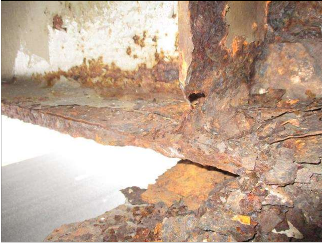
Span 3 Beam 5: BTM FLANGE SECTION LOSS (23% SL, 7/16IN SL, 1/2IN REMAIN) 6IN WIDE AT RIGHT SIDE FOR 1FT AT FAR END. BEARING STIFFENER ON RIGHT SIDE OF BEAM HAS A HOLE FOR UP TO 2 IN HIGH 1 IN WIDE NEAR MID HEIGHT. (PAR)
