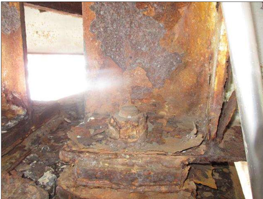
Span 4 Beam 9: WEB SECTION LOSS (9/16IN REMAIN) FULL HEIGHT FOR 19IN AT NEAR END.
