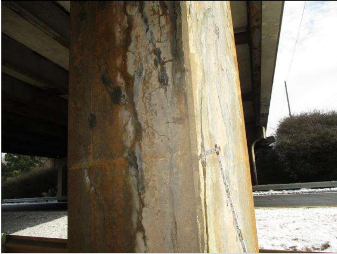
Bent 2 Pile 5: FULL HEIGHT VERTICAL OPEN CRACKING (UP TO 1/2N) TO ALL FACES OF COLUMN & FULL HEIGHT DELAM (12IN WIDE) AT NEAR FACE. ADDITIONAL SPALL IN SOUTH FACE OF PILE UP TO 5 IN LONG X 1 IN DEEP X 1 IN WIDE. (PAR)
