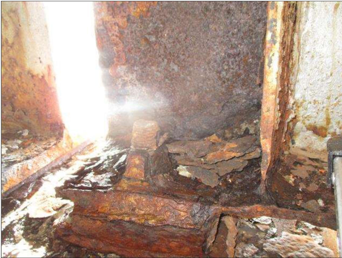
Span 1 Beam 10: BTM FLANGE SECTION LOSS (47% SL, 7/16IN SL, 1/2IN REMAIN) FULL WIDTH & WEB PITTING (1/2IN REMAIN) X 6IN HIGH FOR 4FT AT FAR END. (PAR)
