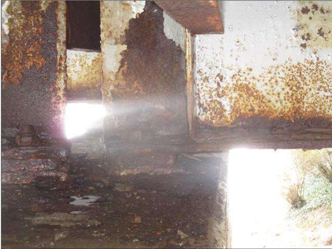
Span 1 Beam 2: BTM FLANGE SECTION LOSS (33% SL, 5/16IN SL, 5/8IN REMAIN) FULL WIDTH & WEB PITTING (9/16IN REMAIN) X 3IN HIGH FOR 2FT AT FAR END. STIFFENER SECTION LOSS (1/4IN REMAIN) 3IN HIGH X 2IN WIDE TO LEFT SIDE STIFFENER AT FAR END. (PAR)
