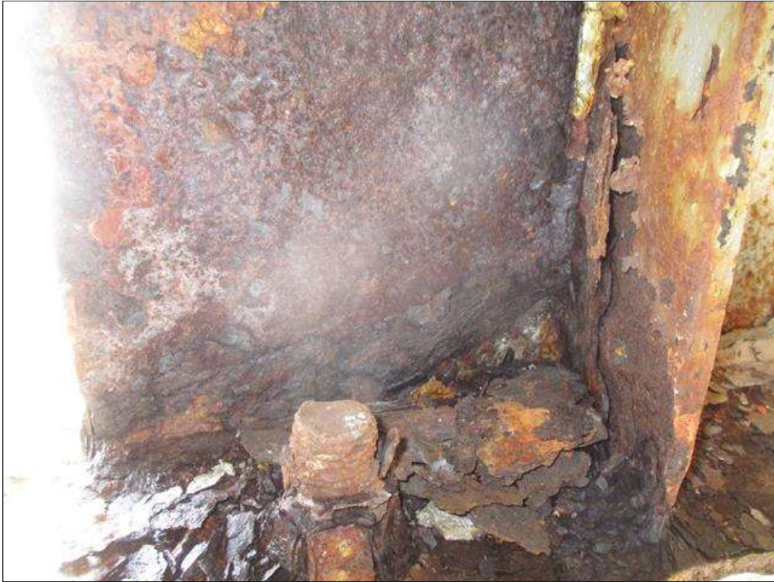
Span 1 Beam 10: WEB SECTION LOSS (3/16IN SL, 7/16 REMAIN) X FULL HEIGHT FOR 8IN AT FAR END. STIFFENER SECTION LOSS (1/4IN REMAIN) 2IN HIGH X 3IN WIDE TO LEFT SIDE STIFFENER AT FAR END. (PAR)
