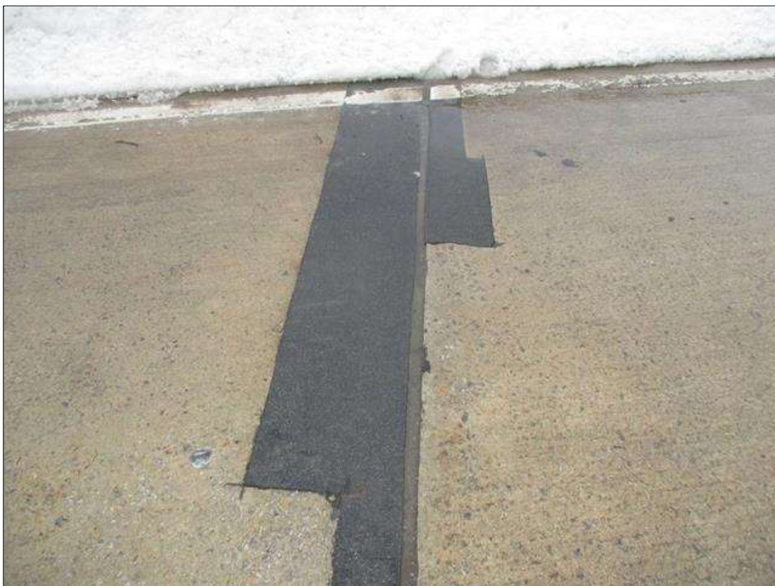
Span 1 Deck: SOUND PATCH (8FT X 2FT) IN LEFT EASTBOUND LANE AT NEAR END AT PREVIOUS: eastbound left lane next to median at end bent 1, broken concrete (8ft x 18in x up to 1/8in) and depressed (1/4in)
