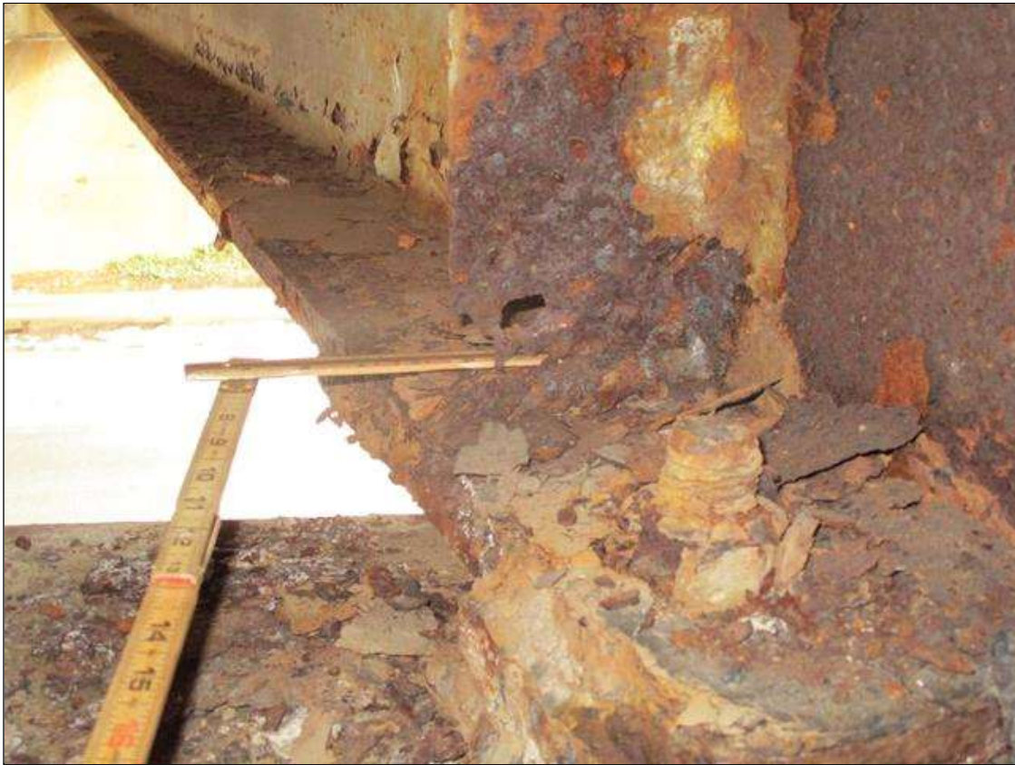
Span 3 Beam 8: WEB SECTION LOSS (UP TO 100% SL AT TOP, AVG. 1/8IN REMAIN) X FULL HEIGHT FOR 10IN AT NEAR END. HOLE IN WEB IS 3 IN LONG X 1.5 IN HIGH NEAR THE TOP OF WEB. STIFFENER SECTION LOSS (UP TO 100%SL, AVG 1/16IN REMAIN) 8IN HIGH X FULL WIDTH TO LEFT SIDE STIFFENER AT NEAR END. HOLE IS 2IN WIDE X 2IN HIGH. STIFFENER SECTION LOSS (1/4IN REMAIN) 8IN HIGH X FULL WIDTH TO RIGHT SIDE STIFFENER AT NEAR END. (PAR)
