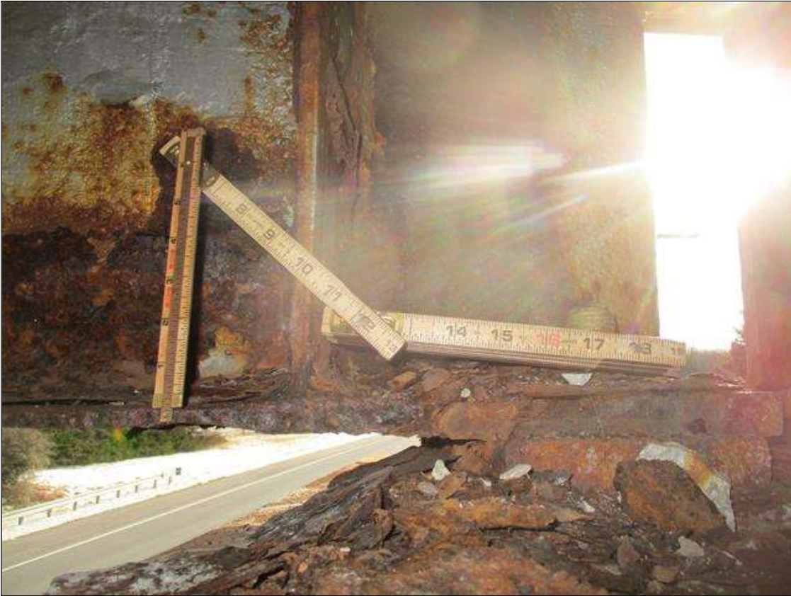
Span 3 Beam 10: BTM FLANGE SECTION LOSS (40% SL, 3/8IN SL, 9/16IN REMAIN) FULL WIDTH & WEB PITTING (1/8IN REMAIN) X FULL HEIGHT FOR 6 INCHES AT NEAR END. (PAR)
