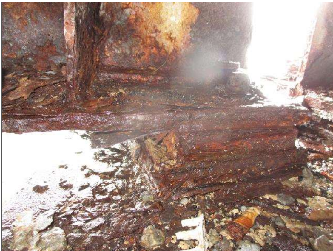
Span 4 Beam 10 - Far Bearing: MODERATE SCALING TO BEARING
