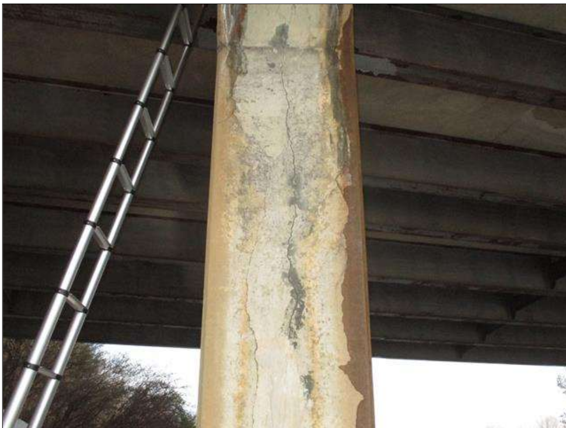
Bent 1 Pile 3: PATCHED AREA UNSOUND ALONG SOUTH FACE FOR 2/3 OF TOTAL HEIGHT
