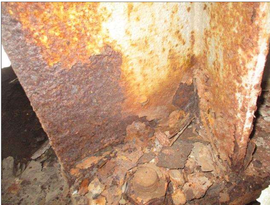
Span 4 Beam 3: WEB SECTION LOSS (40% SL, 1/4IN SL, 3/8IN REMAIN) X UP TO FULL HEIGHT FOR 10IN AT NEAR END. (PAR)
