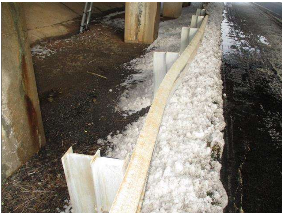
TWO AREAS OF MINOR GUARDRAIL DAMAGE UP TO 10 FT LONG ALONG HIGHWAY 29 SOUTHBOUND LANES RIGHT RAIL.
