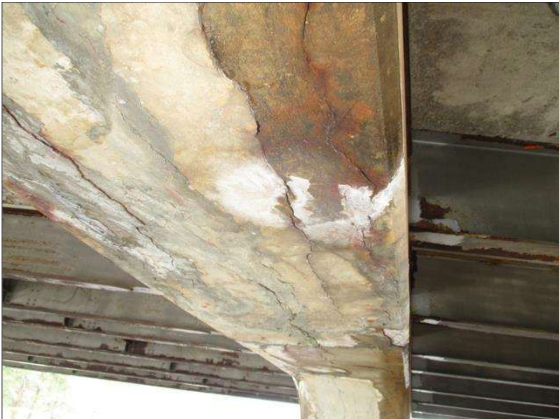
Bent 3 Cap 1: LONGITUDINAL CRACKING UP TO 3/16 IN WIDE WITH SURROUNDING DELAMS ON THE UNDERSIDE OF CAP BETWEEN PILES 3 AND 4
