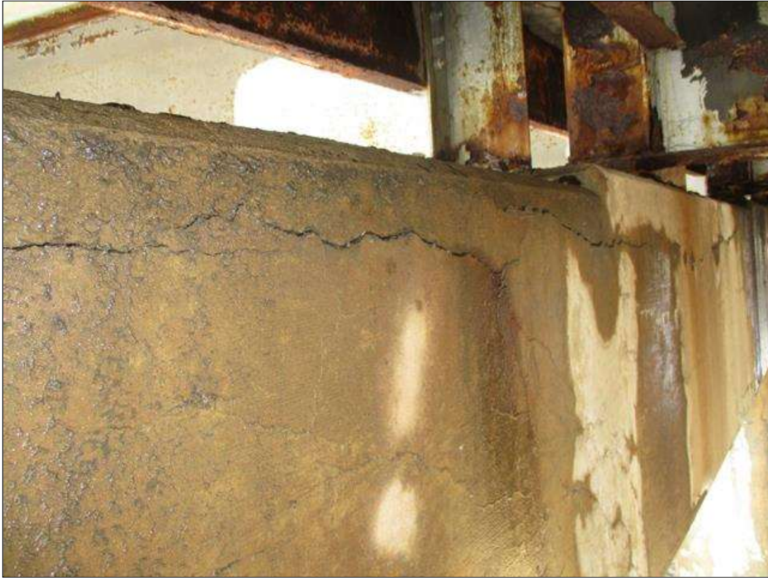
Bent 3 Cap 1: HORZ. & MAP CRACKING (UP TO 3/16IN) WEST/ EFFLO. & RUSTING STAINING THRU OUT ALL FACES OF CAP. HORZ. CRACKING (UP TO 1/8IN) WEST/ EDGE DELAM TO BTM OF CAP THRU OUT.
