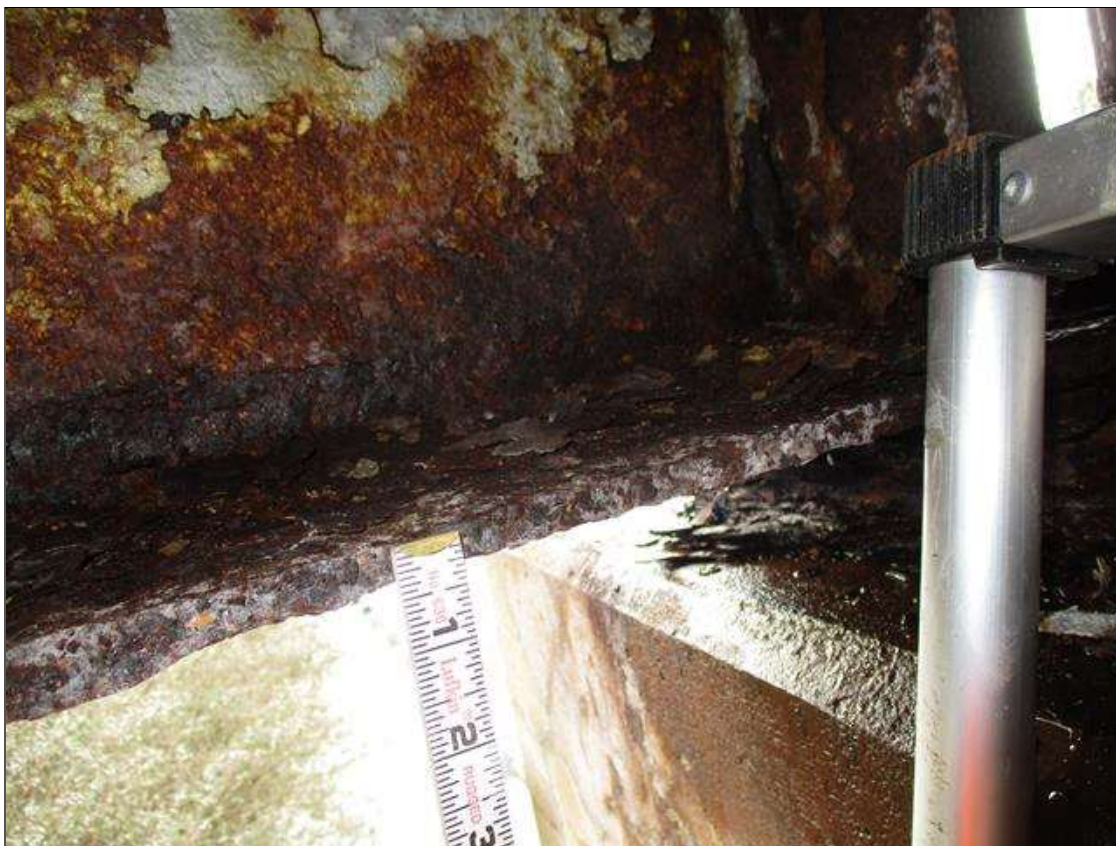
Span 4 Beam 10: BTM FLANGE SECTION LOSS (46% SL, 3/8IN SL, 7/16IN REMAIN) FULL WIDTH & WEB PITTING (9/16IN REMAIN) X 4IN HIGH FOR 4FT AT NEAR END.(PAR)
