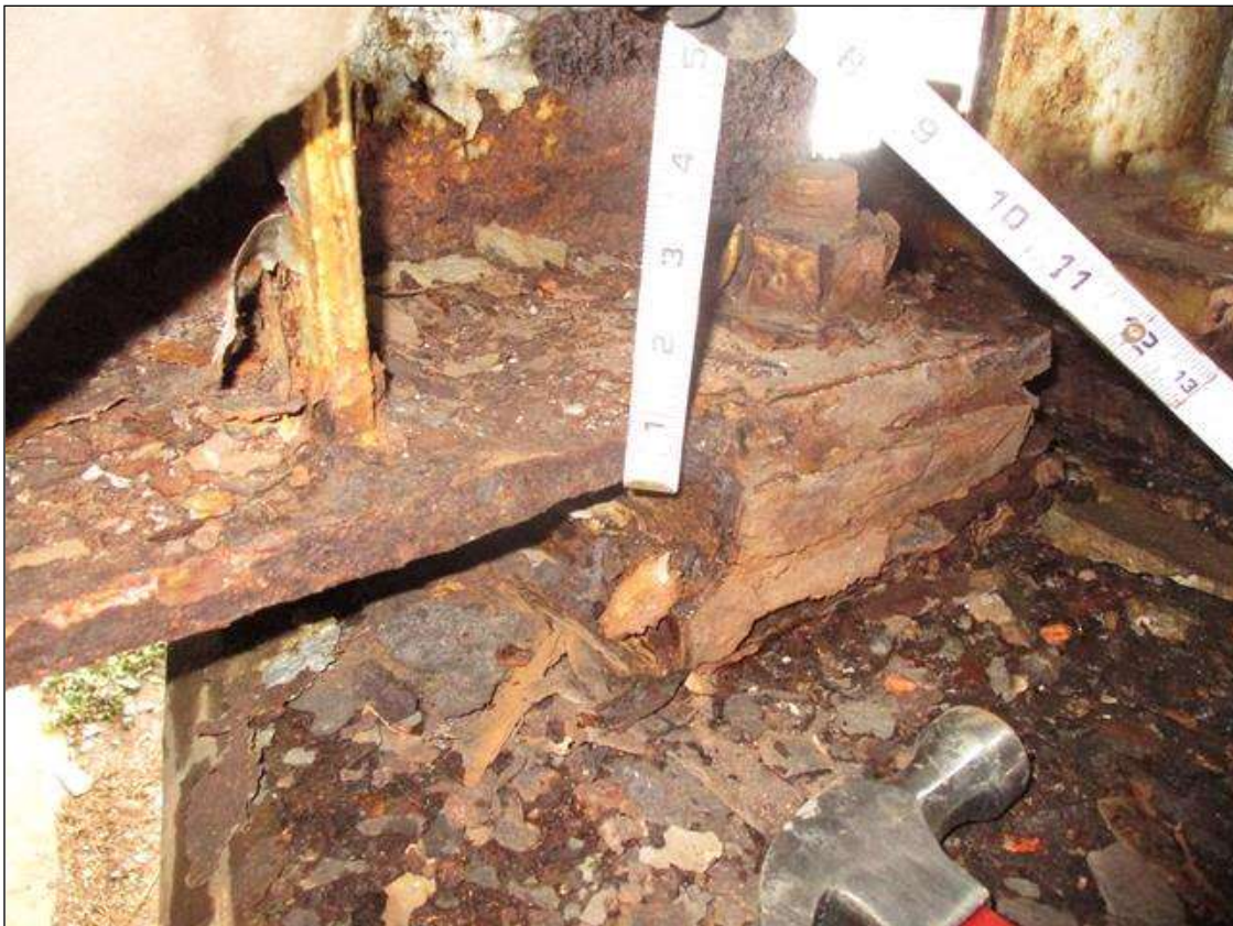
Span 4 Beam 6: BTM FLANGE SECTION LOSS (23% SL, 3/16IN SL, 5/8IN REMAIN) FULL WIDTH FOR 1FT AT NEAR END. (PAR)
