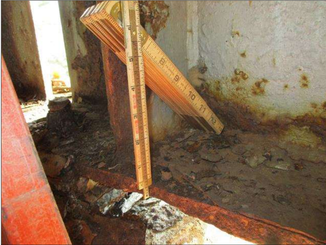
Span 2 Beam 10: BTM FLANGE SECTION LOSS (47% SL, 7/16IN SL, 1/2IN REMAIN) FULL WIDTH & WEB PITTING (1/2IN REMAIN) X UP TO FULL HEIGHT FOR 3.5FT AT FAR END.(PAR)
