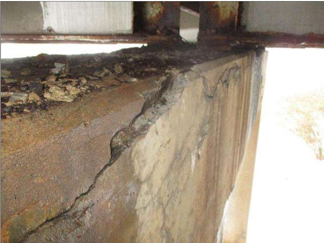
Bent 3 Cap1: DELAMINATED AND SPALLED AREA UP TO 5 FT LONG X 3 HIGH X 2 IN DEEP WITH NO EXPOSED REBAR IN THE TOP FAR FACE BELOW BAY 2 WITH HORIZONTAL CRACKS UP TO 3/16 IN WIDE
