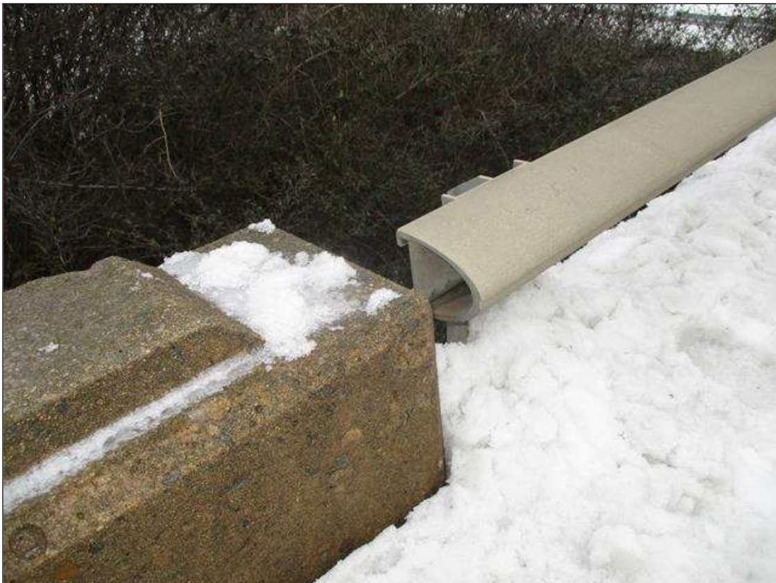
Span 1 Left Bridge Rail: MISSING ALUMINUM END CAP AT NEAR END OF RAIL
