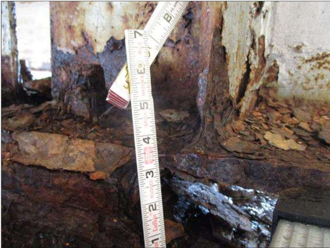
Span 1 Beam 9: BTM FLANGE SECTION LOSS (40% SL, 3/8IN SL, 9/16IN REMAIN) FULL WIDTH FOR 2FT AT FAR END. STIFFENER SECTION LOSS (1/4IN REMAIN) 3IN HIGH X 3IN WIDE TO LEFT SIDE STIFFENER AT FAR END (PAR)
