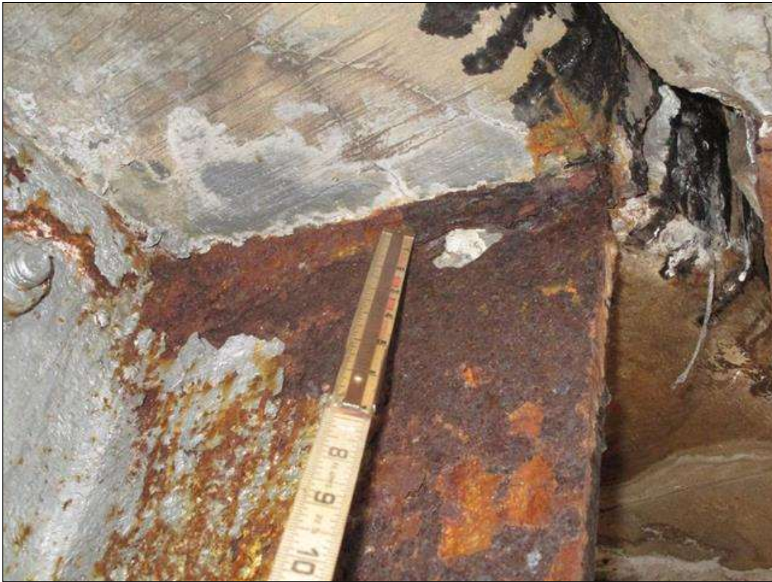
Span 3 Beam 8: WEB SECTION LOSS (UP TO 100% SL AT TOP, AVG. 1/8IN REMAIN) X FULL HEIGHT FOR 10IN AT NEAR END. HOLE IN WEB IS 3 IN LONG X 1.5 IN HIGH NEAR THE TOP OF WEB. STIFFENER SECTION LOSS (UP TO 100%SL, AVG 1/16IN REMAIN) 8IN HIGH X FULL WIDTH TO LEFT SIDE STIFFENER AT NEAR END. HOLE IS 2IN WIDE X 2IN HIGH. STIFFENER SECTION LOSS (1/4IN REMAIN) 8IN HIGH X FULL WIDTH TO RIGHT SIDE STIFFENER AT NEAR END. (PAR)
