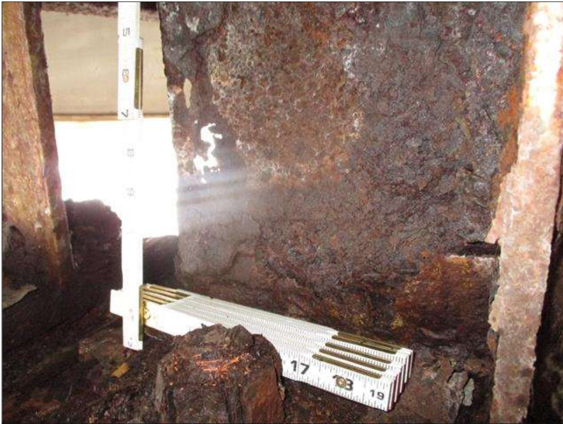
Span 4 Beam 8: WEB SECTION LOSS (UP TO 100% SL, AVG. 1/4IN REMAIN) X FULL HEIGHT FOR 10IN AT NEAR END WITH 3IN HIGH X 2IN LONG HOLE.. STIFFENER SECTION LOSS (UP TO 100%SL, AVG 1/16IN REMAIN) 8IN HIGH X FULL WIDTH TO LEFT SIDE STIFFENER (SIMILAR RIGHT SIDE) AT NEAR END. HOLE IN LEFT STIFFENER IS 2 IN HIGH X 1 IN LONG (PAR).
