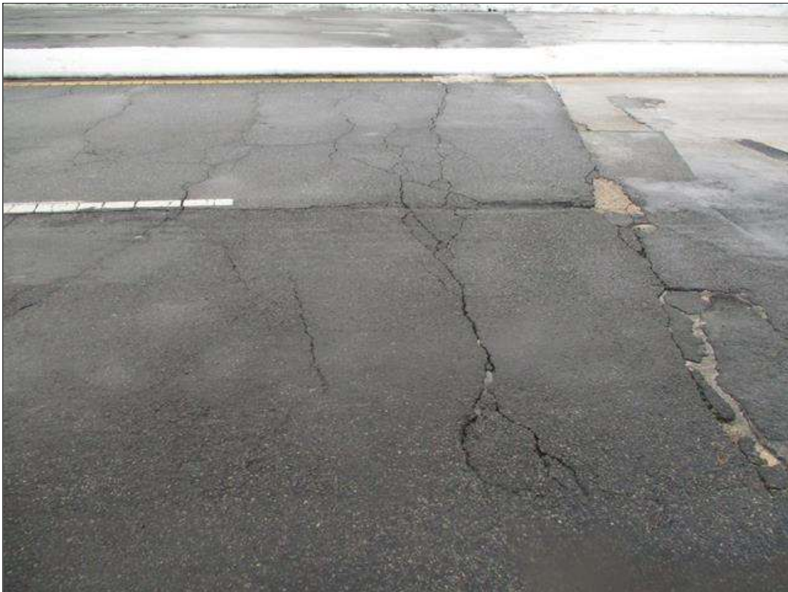
MODERATE SCATTERED CRACKING UP TO 1/2 IN WIDE IN THE APPROACH PAVEMENT NEAR END BENT 2. TYPICAL AT APPROACH PAVEMENT NEAR END BENT 1
