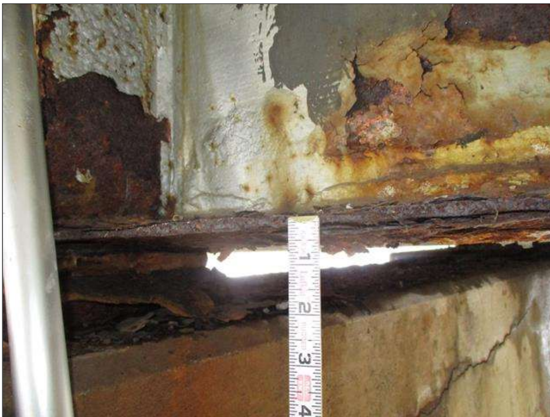
Span 4 Beam 9: BTM FLANGE SECTION LOSS, 3/16IN REMAIN, FULL WIDTH FOR 2FT AT NEAR END. (PAR)
