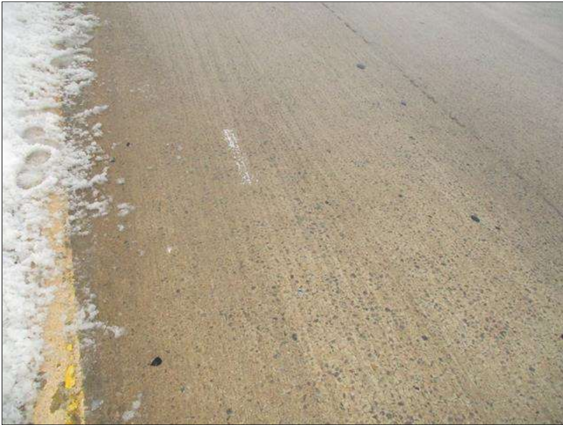
Span 1 Deck: MAP CRACKING (HAIRLINE TO 1/16IN) & WEAR WEST/ EXPOSED AGGREGATE THRU OUT CONCRETE DECK IN TRAVEL LANES.
