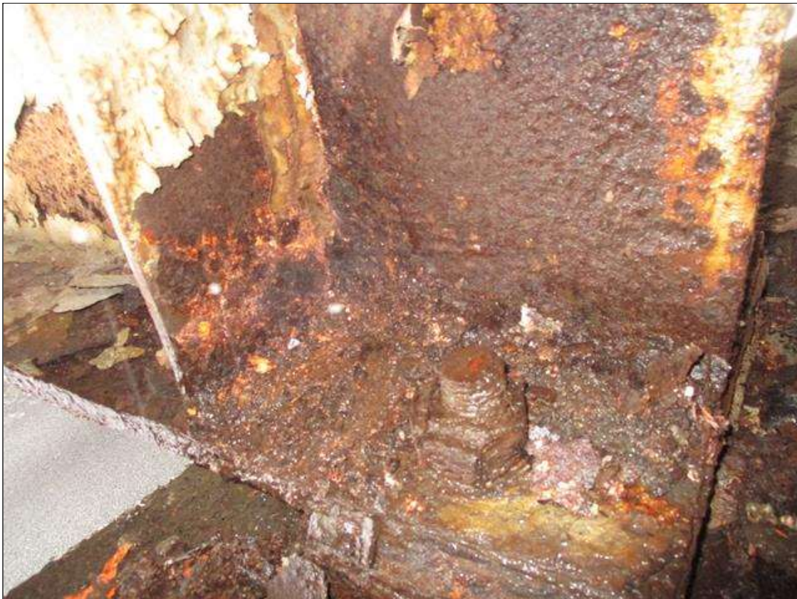
Span 2 Beam 2: BTM FLANGE SECTION LOSS (27% SL, 1/4IN SL, 11/16IN REMAIN) FULL WIDTH FOR 4FT AT NEAR END. WEB SECTION LOSS (1/8IN SL, 1/2IN REMAIN) 2IN HIGH FOR 4IN AT NEAR END. (PAR)
