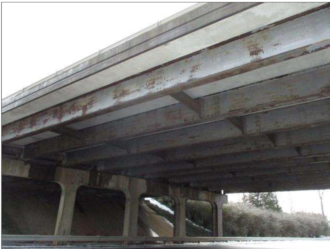
Span 3 Beam 1 - Protective System: AREAS OF PC LOSS THRU OUT LENGTH OF BEAM, MOSLTY AT FLANGES & BEAM ENDS
