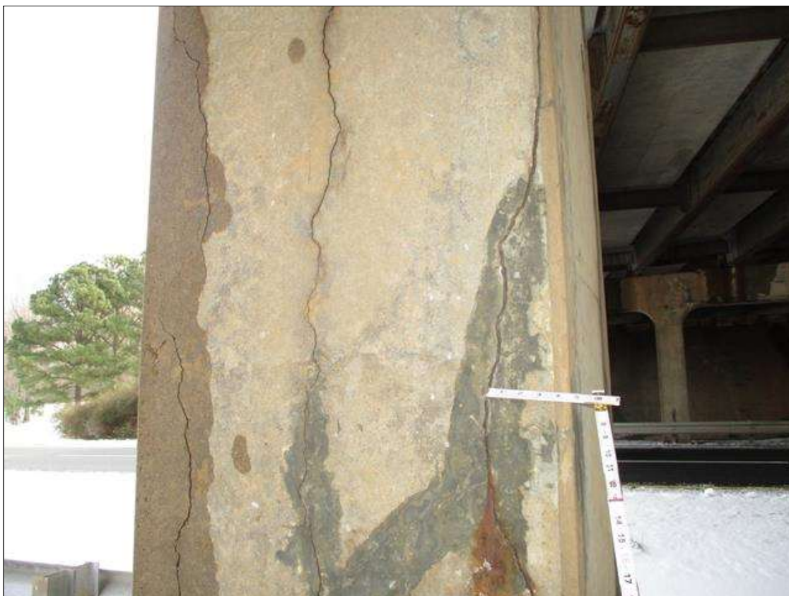
Bent 2 Pile 1: FULL HEIGHT VERTICAL OPEN CRACKING (UP TO 3/16IN) TO ALL FACES OF COLUMN. (PAR)
