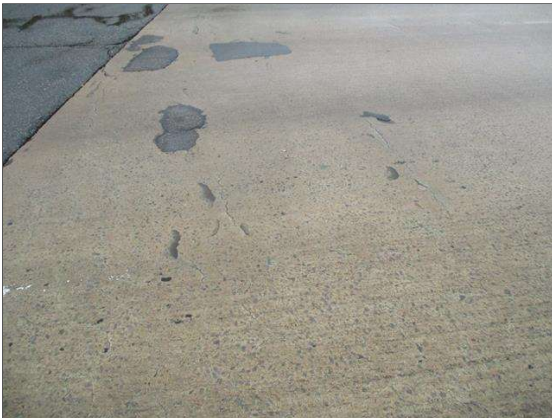
Span 1 Deck: TRANSVERSE OPEN CRACKING (UP TO 1/8IN) THRU OUT CONCRETE DECK IN ALL LANES. DIAGONAL OPEN CRACKING IN LEFT LANES.
