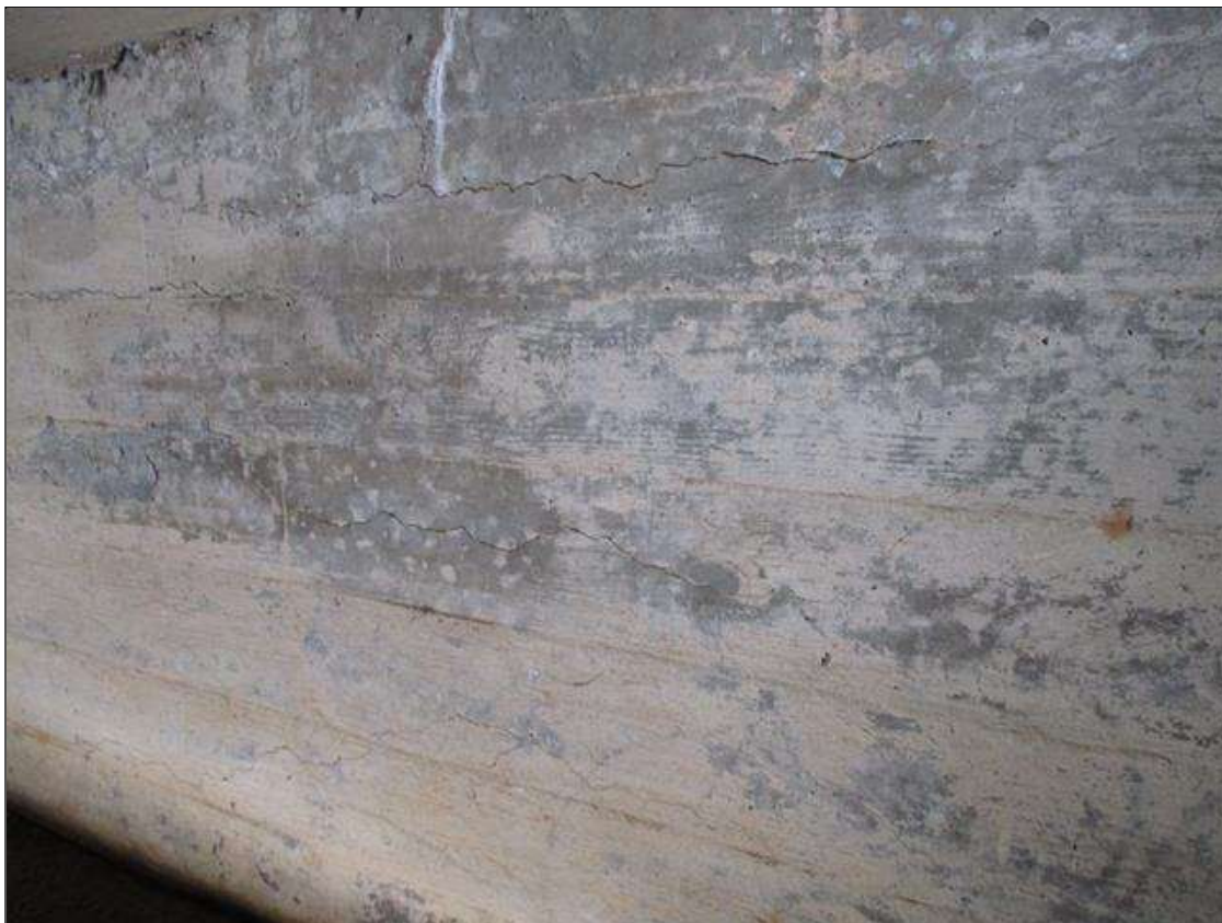
End Bent 2 Abutment: MULTIPLE HORZ. CRACKS UP TO 1/16TH IN WIDE THRU OUT END BENT BACKWALL AT OUTSIDE FACES.
