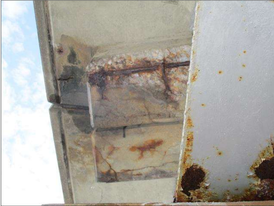
Span 2 Deck: SPALL (2FT X 8IN X 2IN) WEST/ EXPOSED REBAR TO LEFT SIDE OVERHANG HAUNCH OVER BENT 2. UP TO 90% SECTION REMAINING IN THE EXPOSED REBAR (PAR)
