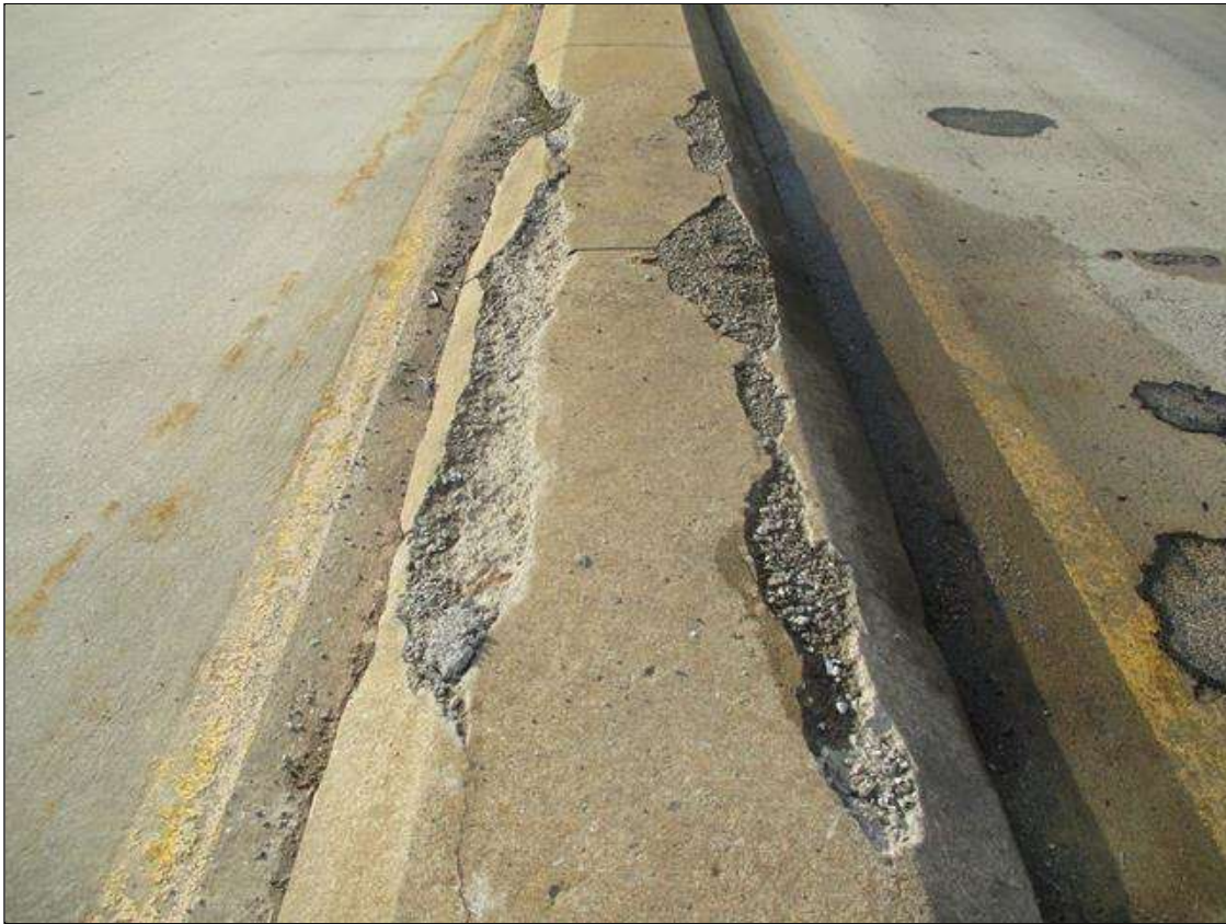
Span 2 Deck: 2X SPALLING (UP TO 17FT X 1FT WIDE X 6IN) DEEP TO RIGHT & LEFT SIDES OF MEDIAN AT FAR END. SPALL (2FT X 10IN X 6IN DEEP) TO RIGHT SIDE OF MEDIAN AT 1/3 SPAN (SIMILAR AT 2/3 SPAN).
