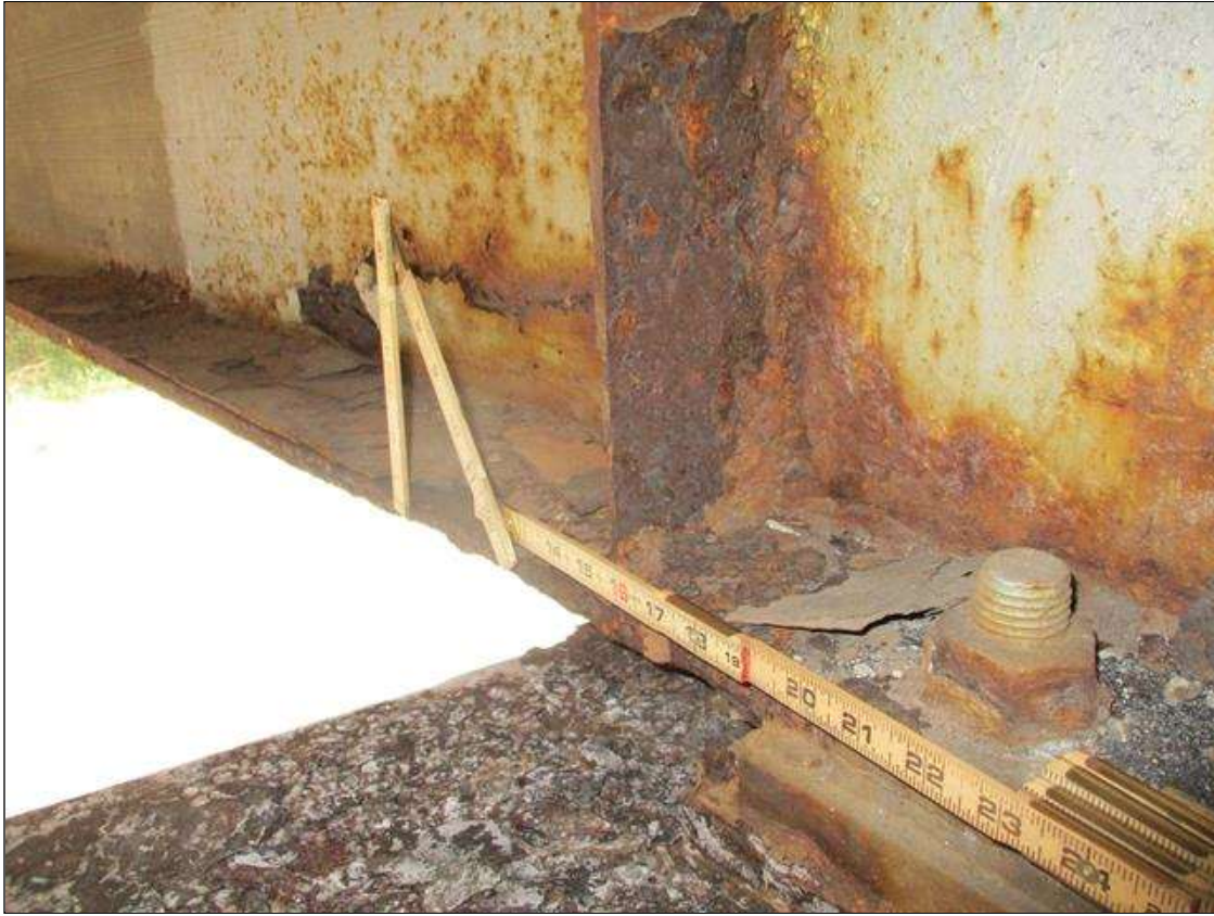
Span 3 Beam 9: BTM FLANGE SECTION LOSS (47% SL, 7/16IN SL, 1/2IN REMAIN) FULL WIDTH & WEB PITTING (9/16IN REMAIN) X 3IN HIGH FOR 4FT AT NEAR END. STIFFENER SECTION LOSS (1/4IN REMAIN) 8IN HIGH X FULL WIDTH TO LEFT SIDE STIFFENER AT NEAR END (PAR)
