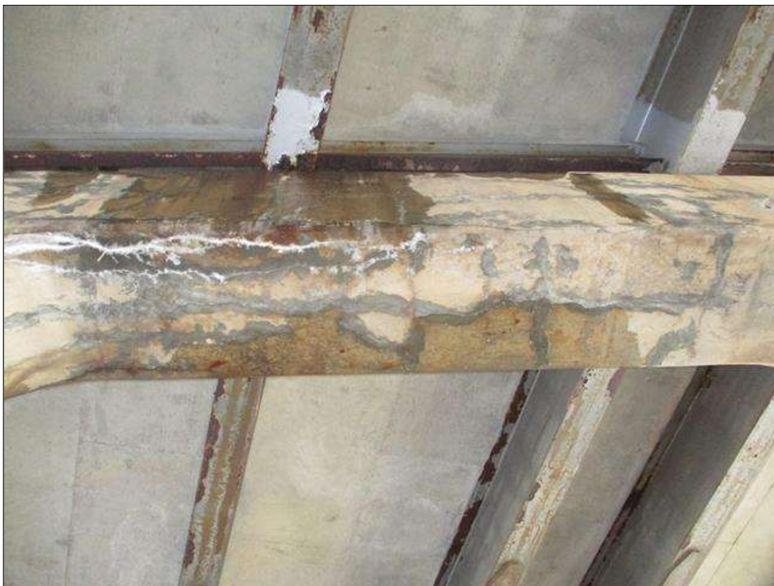
Bent 2 Cap 1: ACTIVE LEAKAGE AT BENT 2 THROUGHOUT LENGTH. TYPICAL AT ALL BENTS
