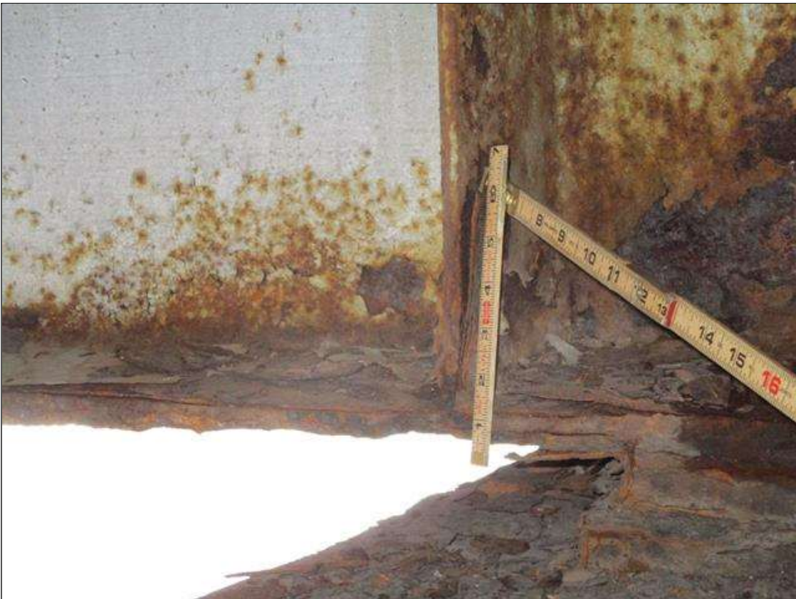
Span 3 Beam 6: BTM FLANGE SECTION LOSS (47% SL, 7/16IN SL, 1/2IN REMAIN) FULL WIDTH FOR 1.5FT AT NEAR END. (PAR)
