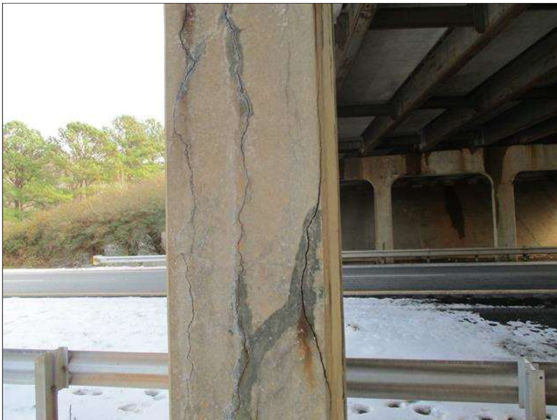
Bent 2 Pile 1: FULL HEIGHT VERTICAL OPEN CRACKING (UP TO 3/16IN) TO ALL FACES OF COLUMN.
