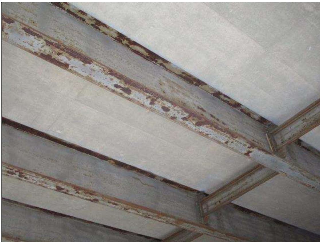
Span 1 Beam 2: SURFACE CORROSION & FRECKLE RUST THRU OUT LENGTH OF BEAM, MOSTLY AT FLANGES.
