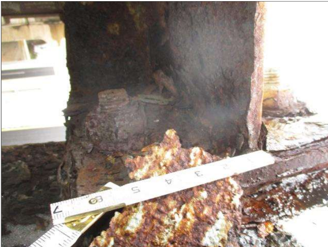
Span 3 Beam 1: BTM FLANGE SECTION LOSS (40% SL, 3/8IN SL, 9/16IN REMAIN) FULL WIDTH FOR 4FT AT FAR END. WEB SECTION LOSS (30% SL, 3/16IN SL, 7/16IN REMAIN) X 10IN HIGH FOR 10IN AT FAR END. (PAR)
