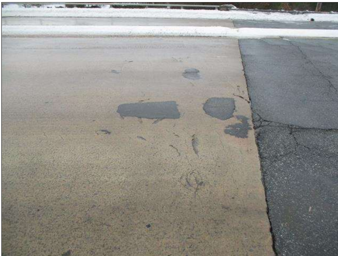
Span 1 Deck: SOUND PATCHES (UP TO 9SQFT) THRU OUT DECK IN BOTH LANES, MOSLTY AT NEAR & FAR ENDS.
