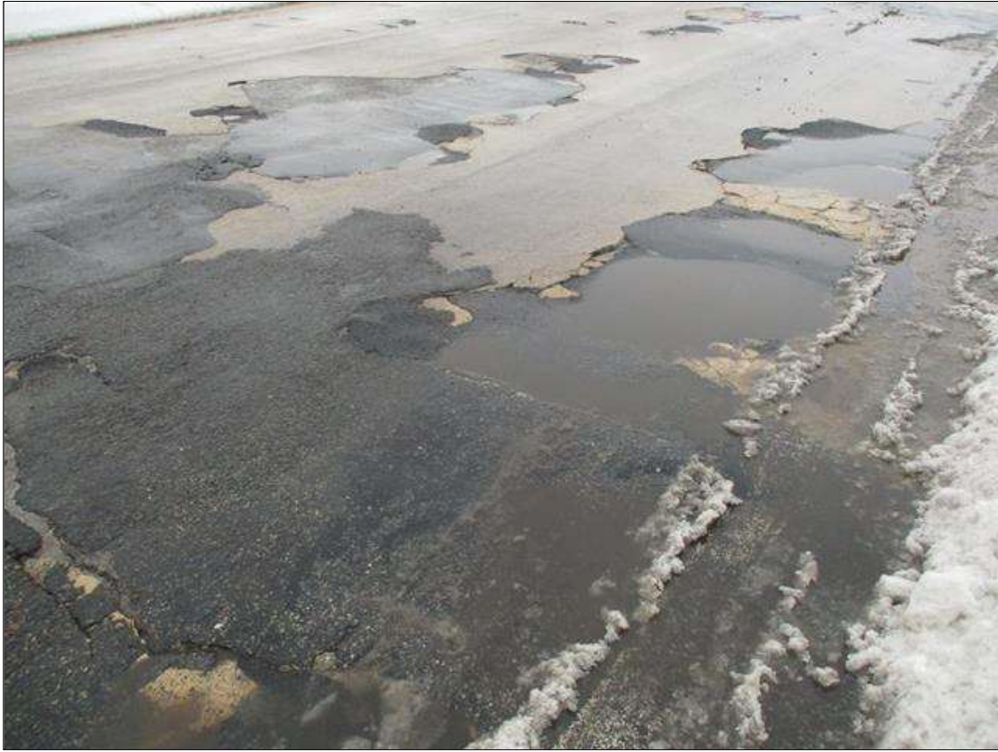
Span 4 Deck: SPALLS UP TO 6 SQ FT WITH PONDING WATER 1 IN DEEP IN RIGHT TRAVEL LANE OF WEST BOUND SIDE FOR FULL LENGTH
