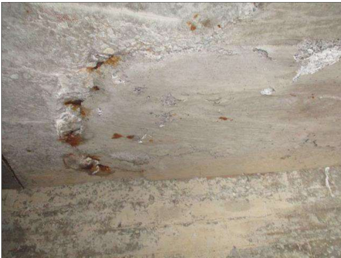
Span 4 Deck: 5 SQ FT AREA OF POORLY PATCHED AREA UNDER BAY 1 WITH SPALLS UP TO 4 IN DIAMETER WITH EXPOSED REBAR. NO SECTION LOSS IN THE EXPOSED REBAR.
