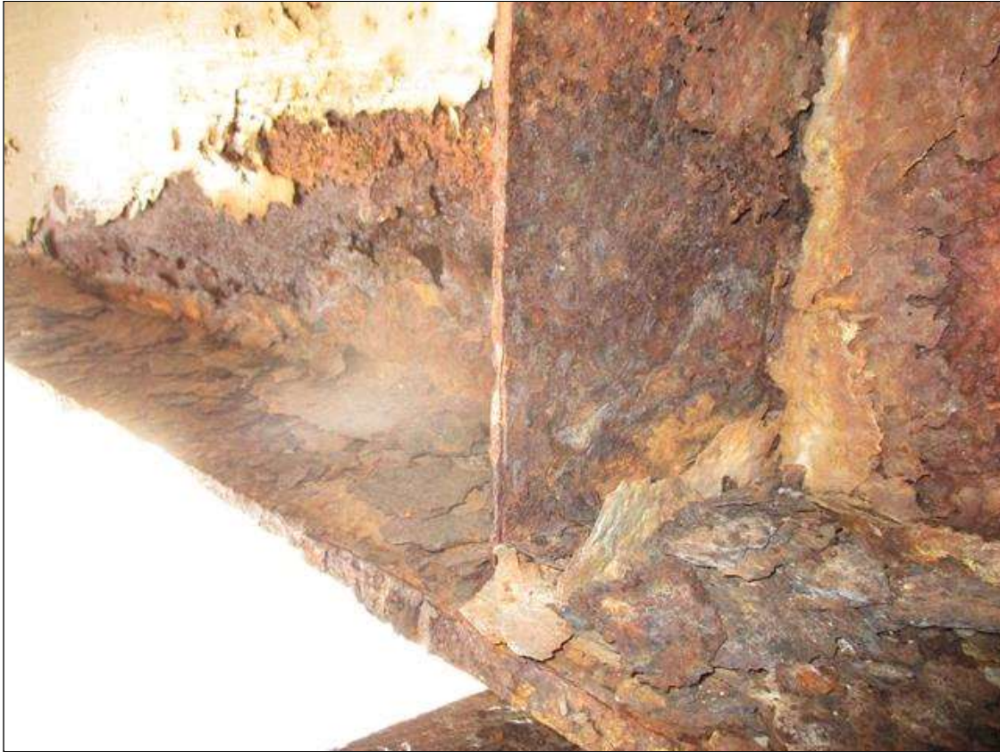
Span 2 Beam 9: BTM FLANGE SECTION LOSS (50% SL, 1/4IN REMAIN AT LEFT SIDE & 1/2IN REMAIN AT RIGHT SIDE) & WEB SECTION LOSS (1/2IN REMAIN) X 8IN HIGH FOR 4FT AT NEAR END. STIFFENER SECTION LOSS (1/4IN REMAIN) 7IN HIGH X FULL WIDTH TO LEFT SIDE STIFFENER AT NEAR END (PAR)
