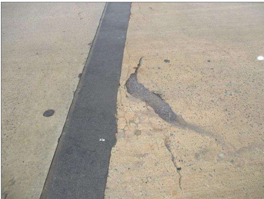
Span 3 Deck: DELAMINATED CONCRETE UP TO 3 FT DIAMETER IN EAST BOUND RIGHT LANE
