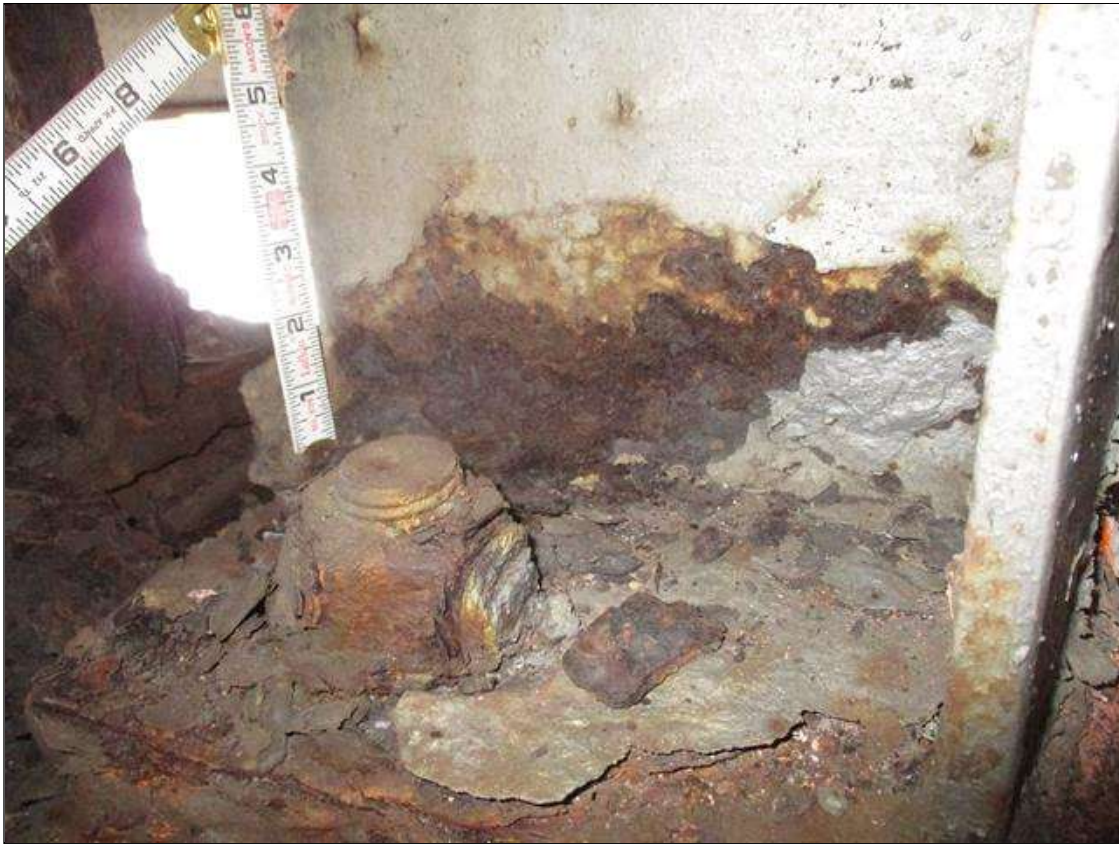
Span 4 Beam 5: SECTION LOSS UP TO 1/8TH IN FOR 6 IN LONG X 10 IN HIGH
