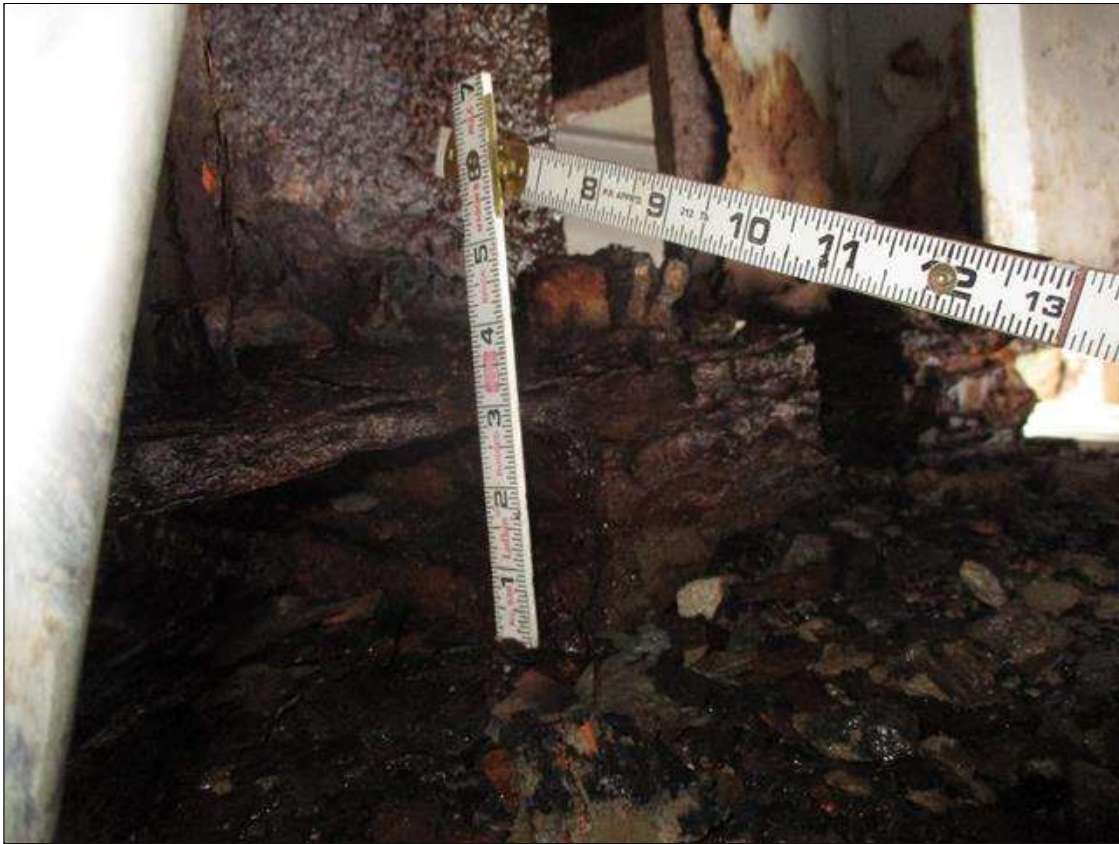
Span 4 Beam 4: BTM FLANGE SECTION LOSS 3/16IN REMAIN, FULL WIDTH FOR 1.5FT AT NEAR END. (PAR)
