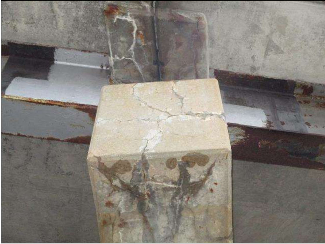
Span 4 Deck: 2X SPALL (UP TO 1.5FT X 8IN X 3IN) WEST/ EXPOSED REBAR TO LEFT SIDE OVERHANG HAUNCH & BTM OF DECK OVER BENT 3. 90% SECTION REMAINING IN THE EXPOSED REBAR. (PAR)
