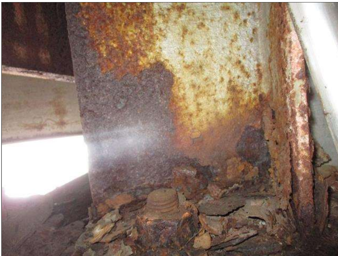
Span 4 Beam 2: BTM FLANGE & FULL HEIGHT WEB SCALING AT NEAR END OF BEAM
