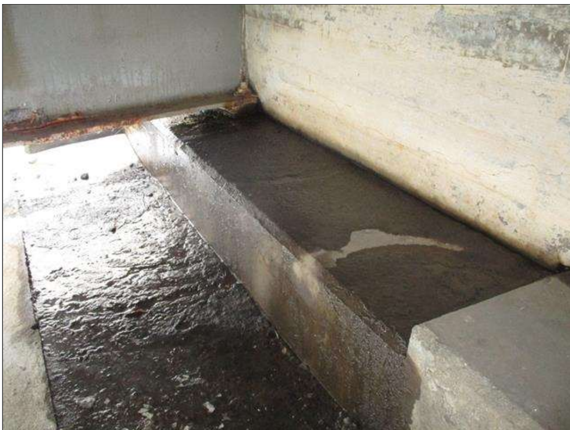
ACTIVE WATER LEAKAGE ON TOP OF BRIDGE SEAT AT BEAM 1 SPAN 4 AT END BENT 2
