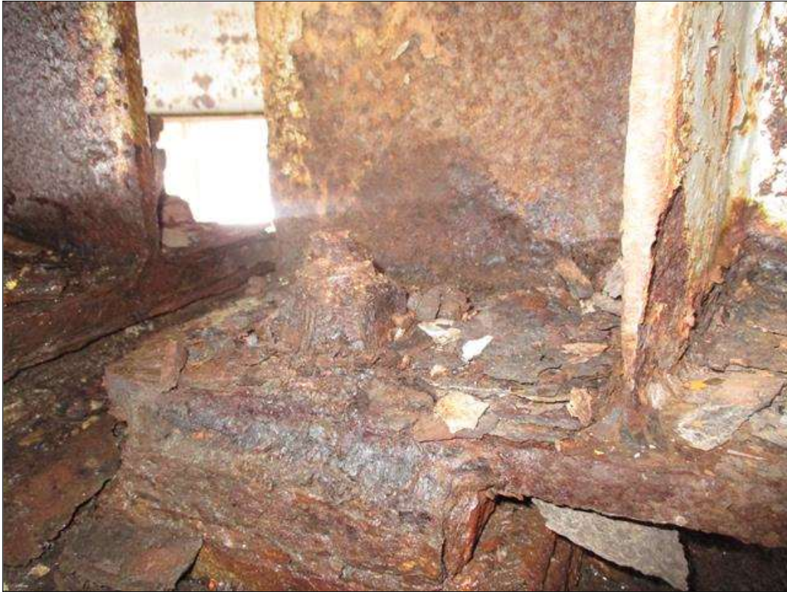
Span 1 Beam 2: BTM FLANGE SECTION LOSS (33% SL, 5/16IN SL, 5/8IN REMAIN) FULL WIDTH & WEB PITTING (9/16IN REMAIN) X 3IN HIGH FOR 2FT AT FAR END. STIFFENER SECTION LOSS (1/4IN REMAIN) 3IN HIGH X 2IN WIDE TO LEFT SIDE STIFFENER AT FAR END. (PAR)
