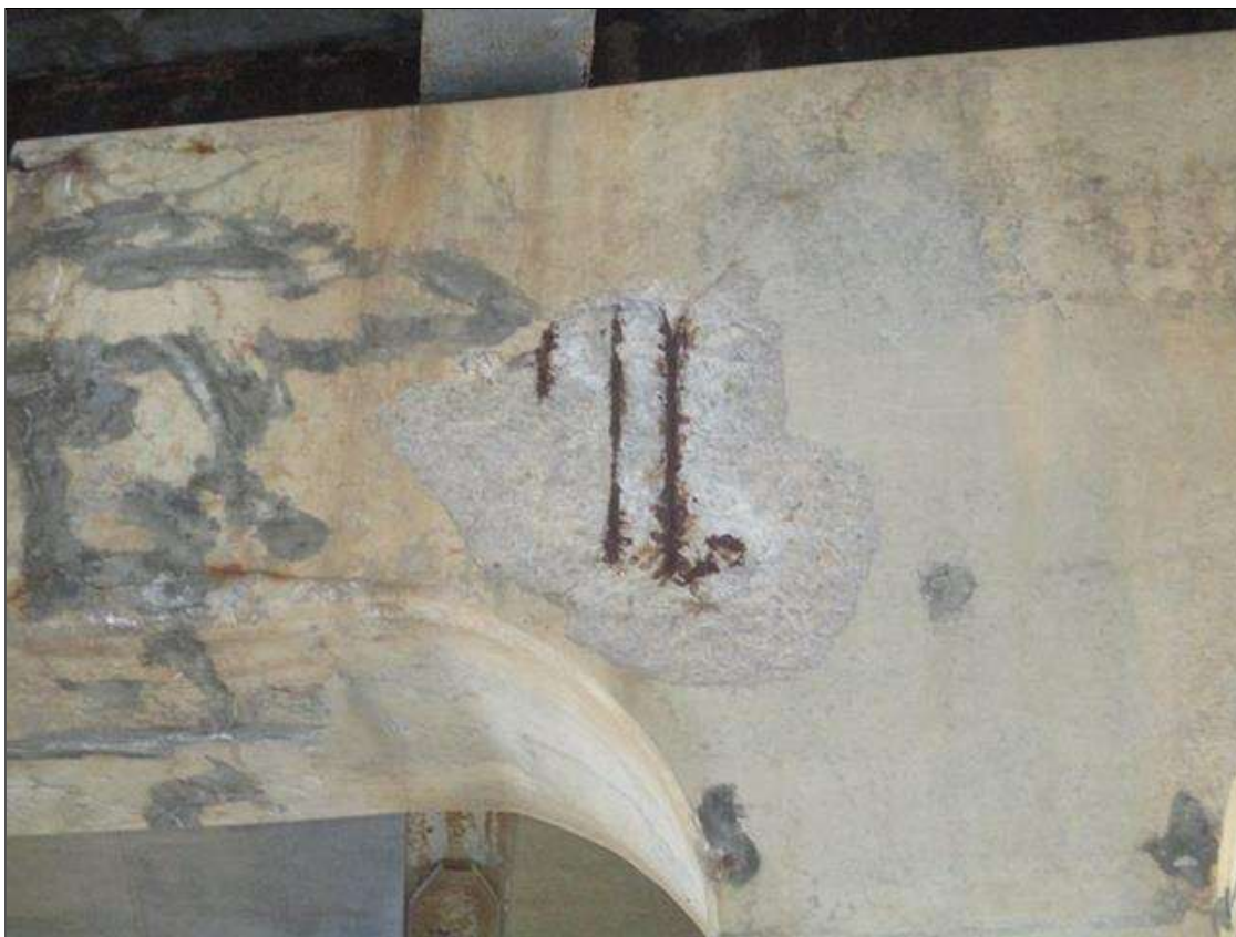
Bent 2 Cap 1: SPALL (3FT X 2FT X 2IN) WEST/ EXPOSED REBAR TO NEAR FACE OF COLUMN OVER COLUMN 3 (PAR)
