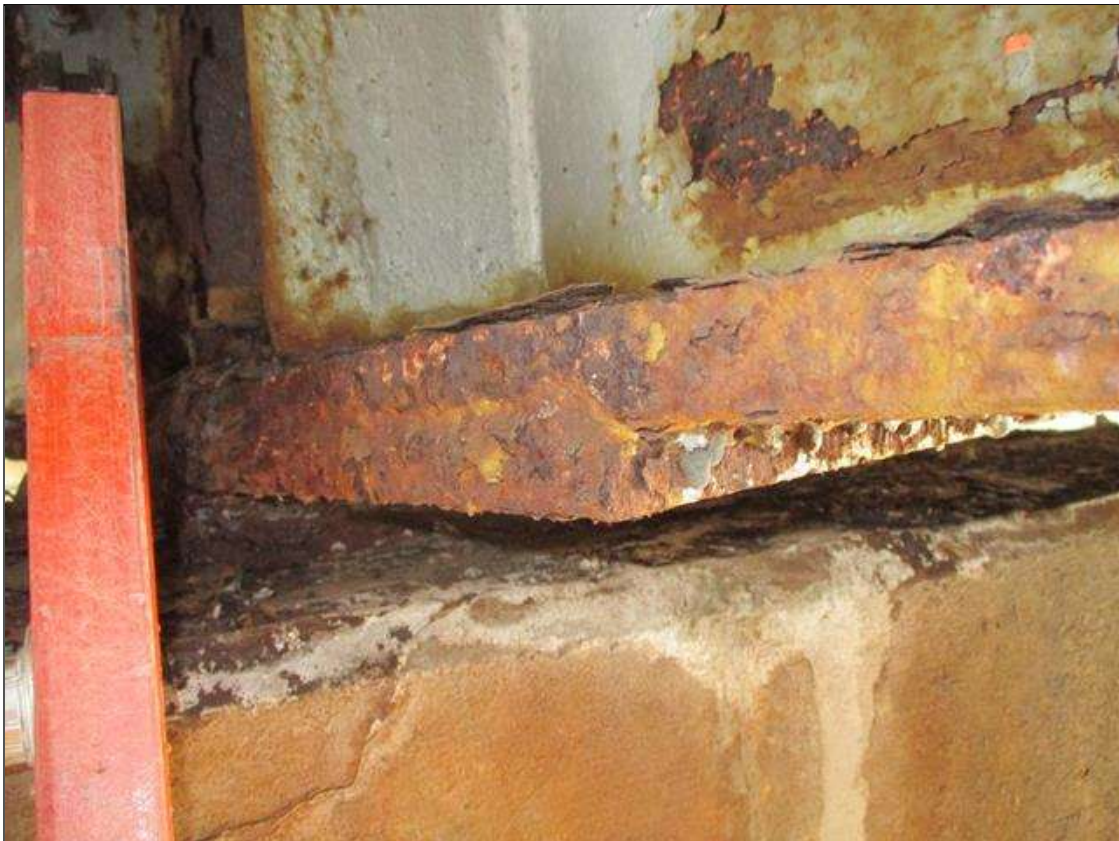
Span 2 Beam 8: BTM MINOR FLANGE SECTION LOSS IS FULL WIDTH FOR 1FT STARTING AT 1FT FROM FAR END AFTER REPAIR PLATE.
