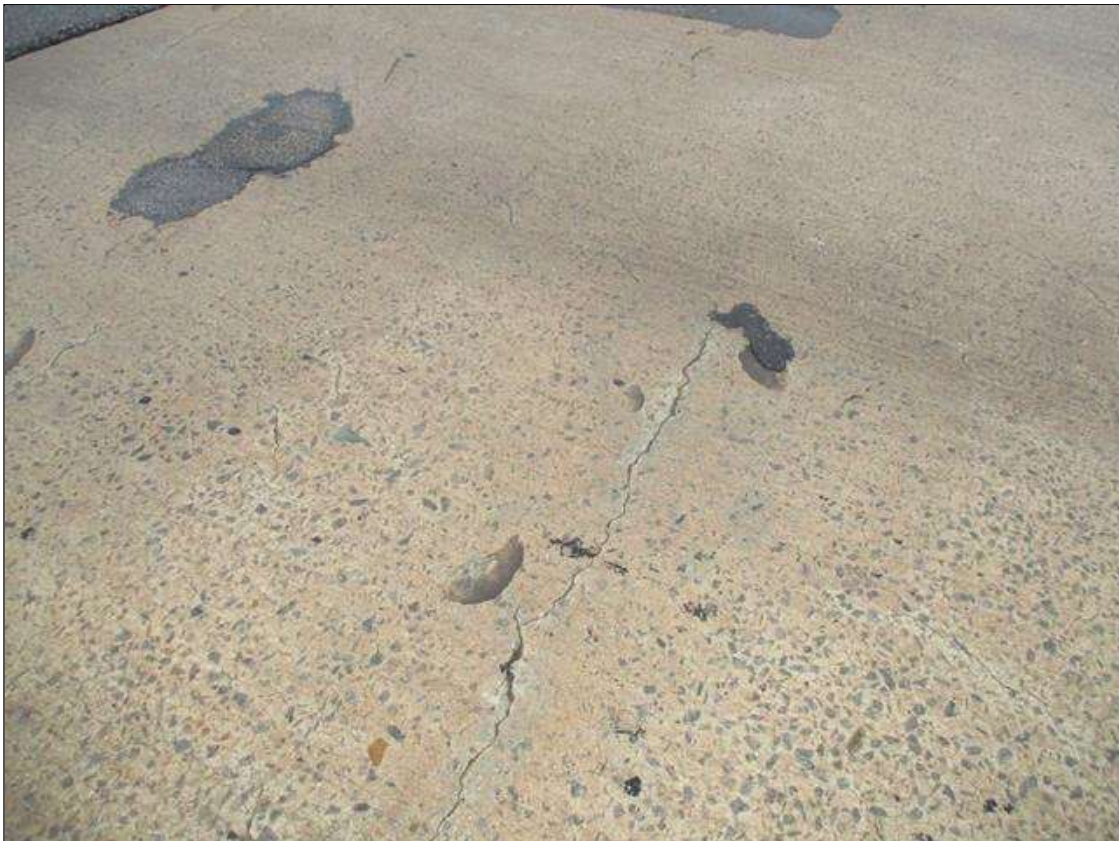
Span 1 Deck: INTERMITTENT SHALLOW SPALLS (UP TO 1.5SQFT X 1/2IN TO 3/4IN DEEP) THRU OUT TOP OF DECK AND AT PERIMETER OF PATCHED AREAS.
