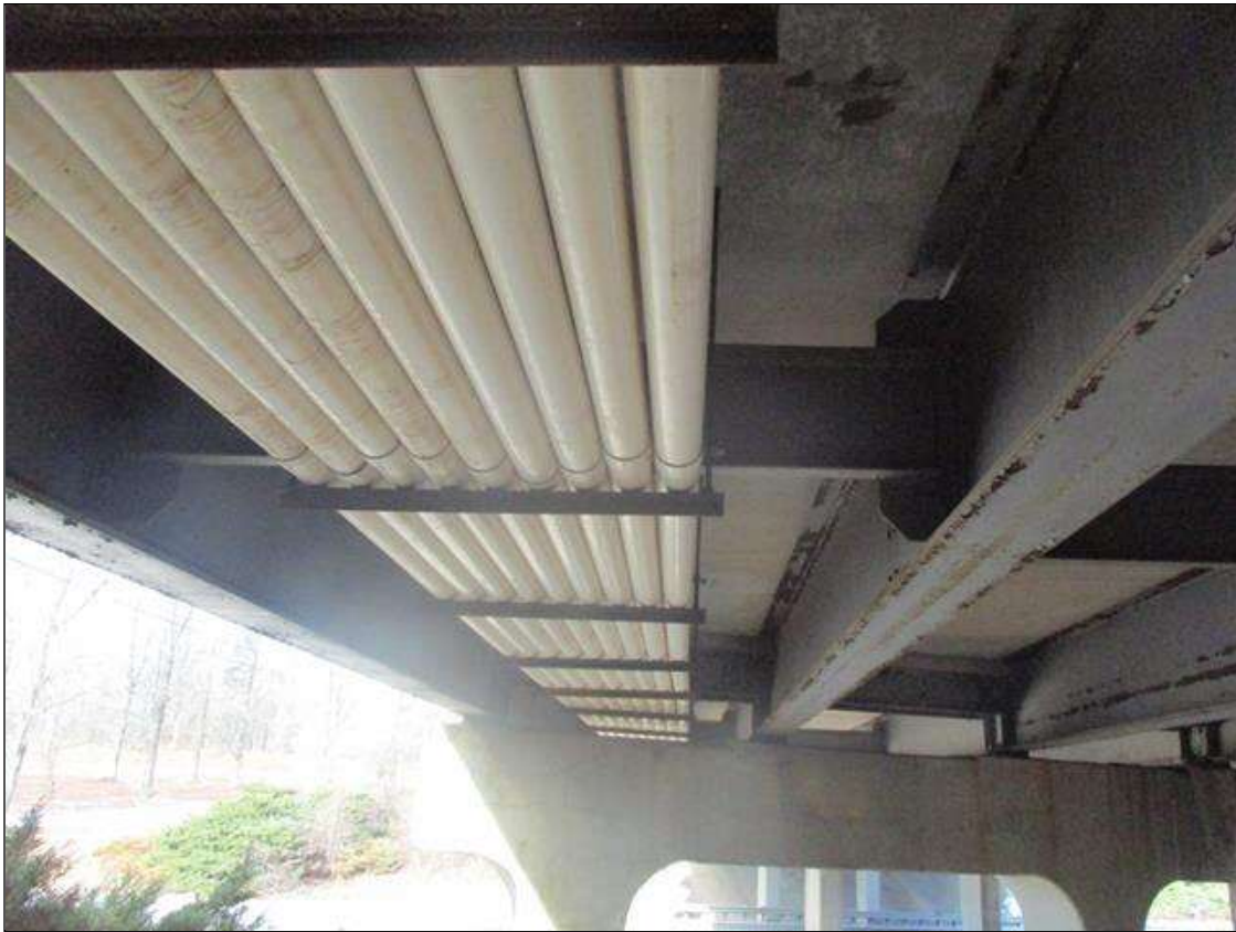
UTILITIES IN BAY 9
