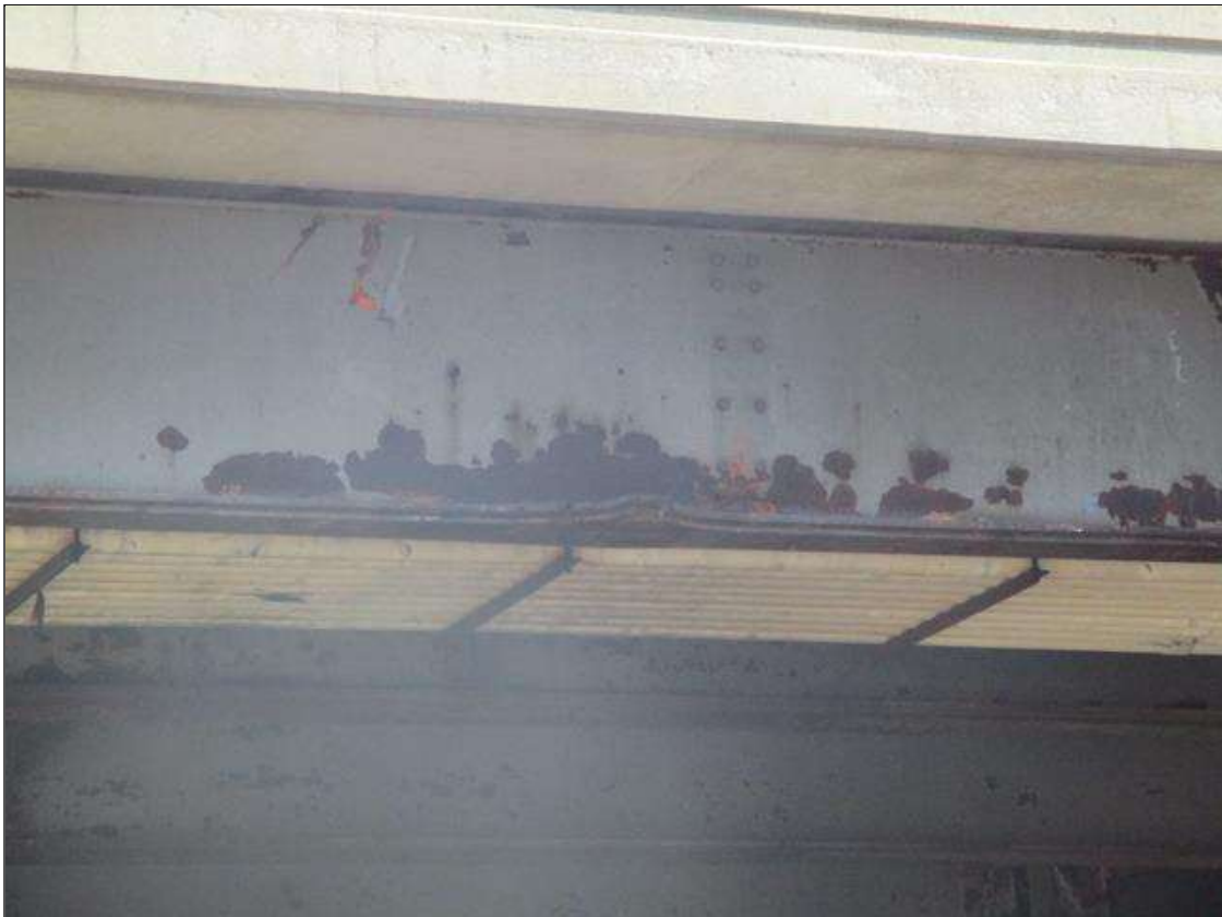
Span 3 Beam 10: IMPACT DAMAGE: 18"L SECTION OF BOTTOM FLANGE AND COVER PLATE BENT UPWARD UP TO 2-1/4" AT 24' FROM BENT 3 BEARING. (PAR)
