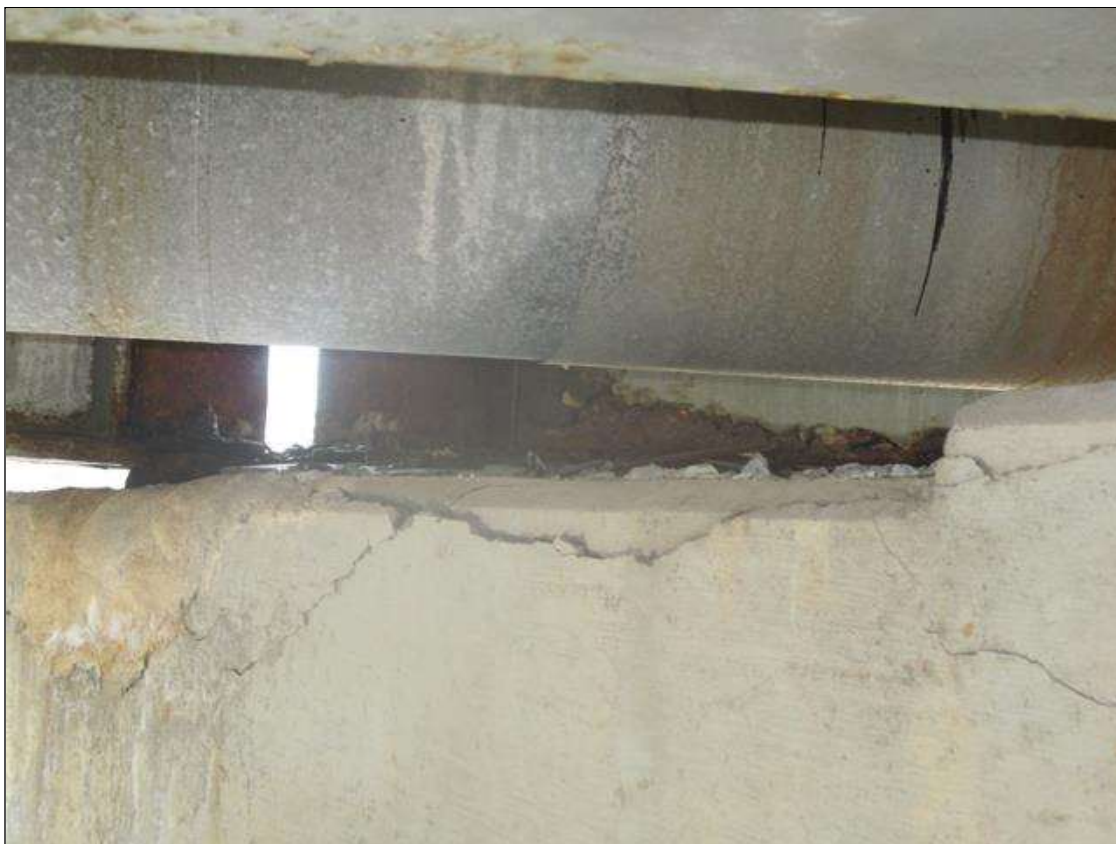
Bent 1 Cap 1: DELAMINATED PATCH (2SF) TO TOP EDGE RIGHT OF BEAM 1, NEAR FACE LEFT END
