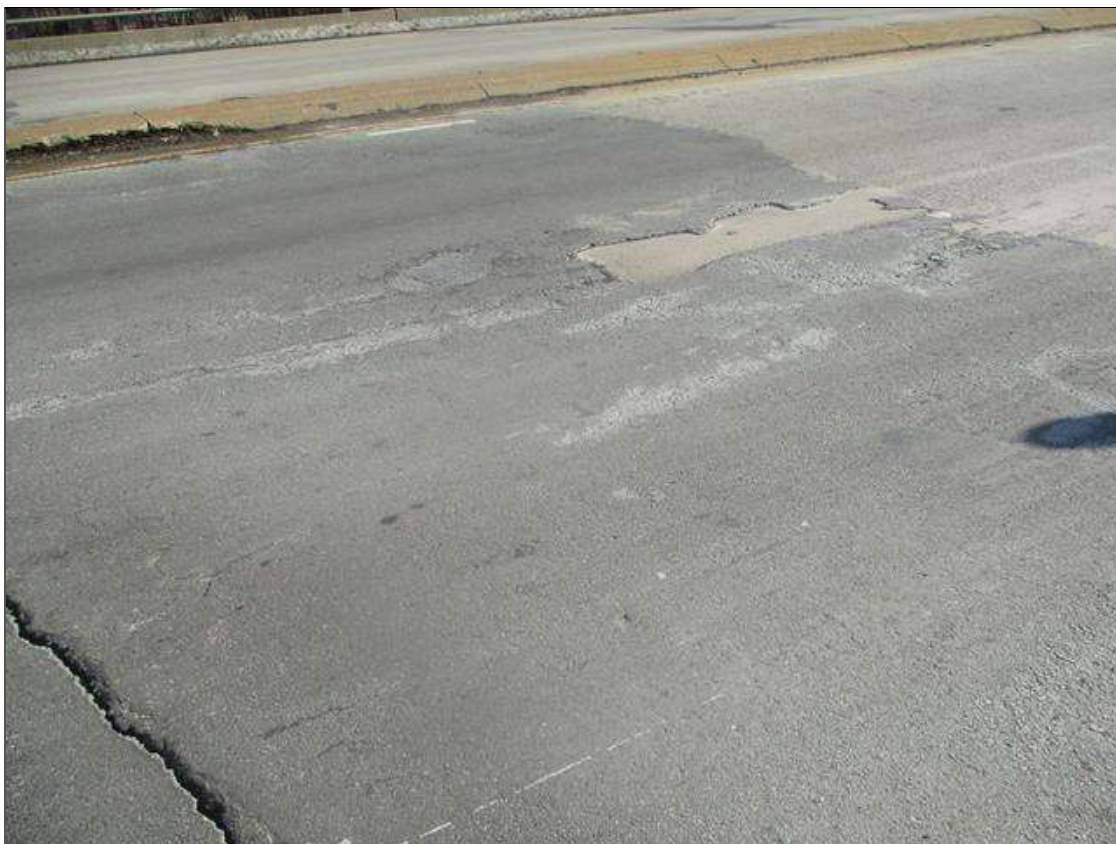
NEW OVERLAY HAS BEEN POURED FOR UP TO 15 FT LONG IN SPAN 1 STARTING AT END BENT 1. HAS MAP CRACKING UP TO 1/16 IN WIDE SCATTERED THOUGHOUT
