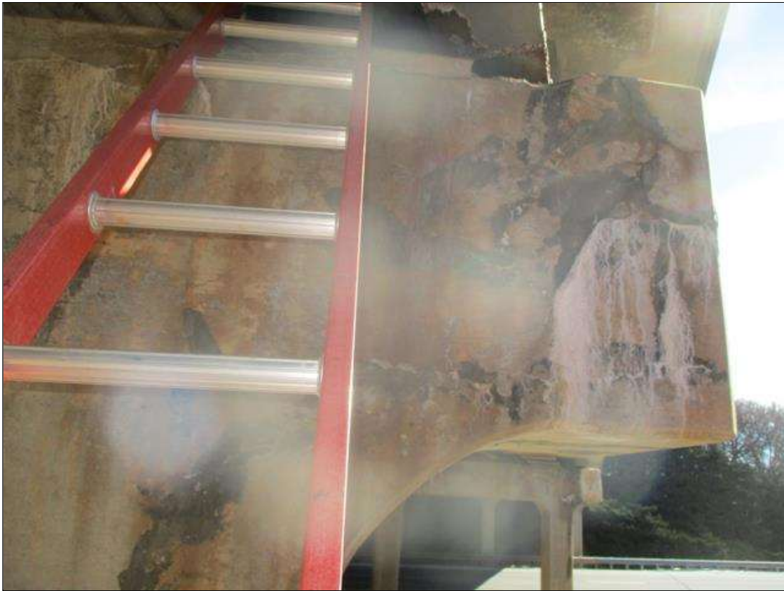
Bent 1 Cap 1: VERTICAL & HORIZONTAL OPEN CRACKING (UP TO 1/16IN X FULL HT.) WITH EFFLO. & RUST STAINING & VERTICAL & HORIZONTAL OPEN CRACKING (UP TO 1/16IN X FULL HT.) WITH EFFLO. & RUST STAINING, NEAR FACE AT RIGHT END
