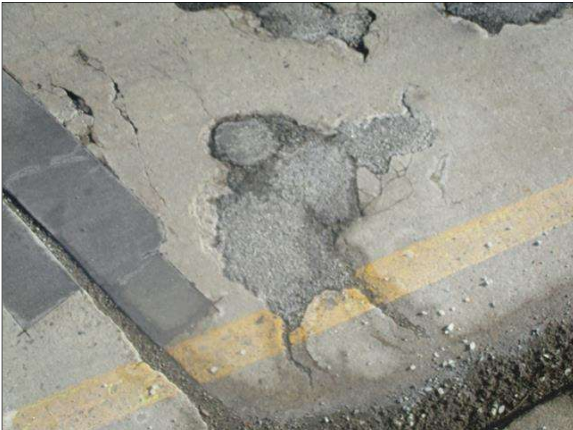
Span 2 Deck: SPALL (12IN X 10IN X 2IN) WITH EXPOSED REINFORCING, NEAR END RIGHT SIDE OF LEFT LANES. - REPAIRED SINCE PREVIOUS INSPECTION. NEW REPAIR
