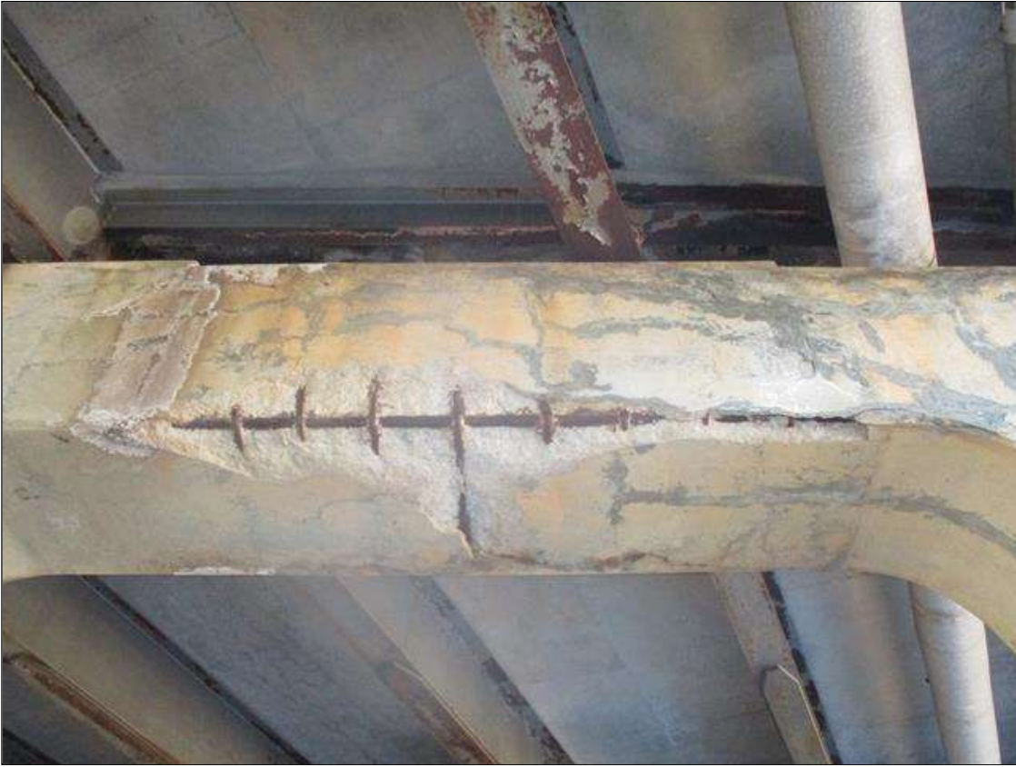
Bent 2 Cap 1: SPALLING (14FT L. X 3FT WIDE X 6IN D.) WITH EXPOSED REINFORCING, TO BOTTOM EDGE & UNDERSIDE AT BEAM 2, FAR FACE. UP TO 90% SECTION REMAINING IN THE EXPOSED REBAR (PAR)
