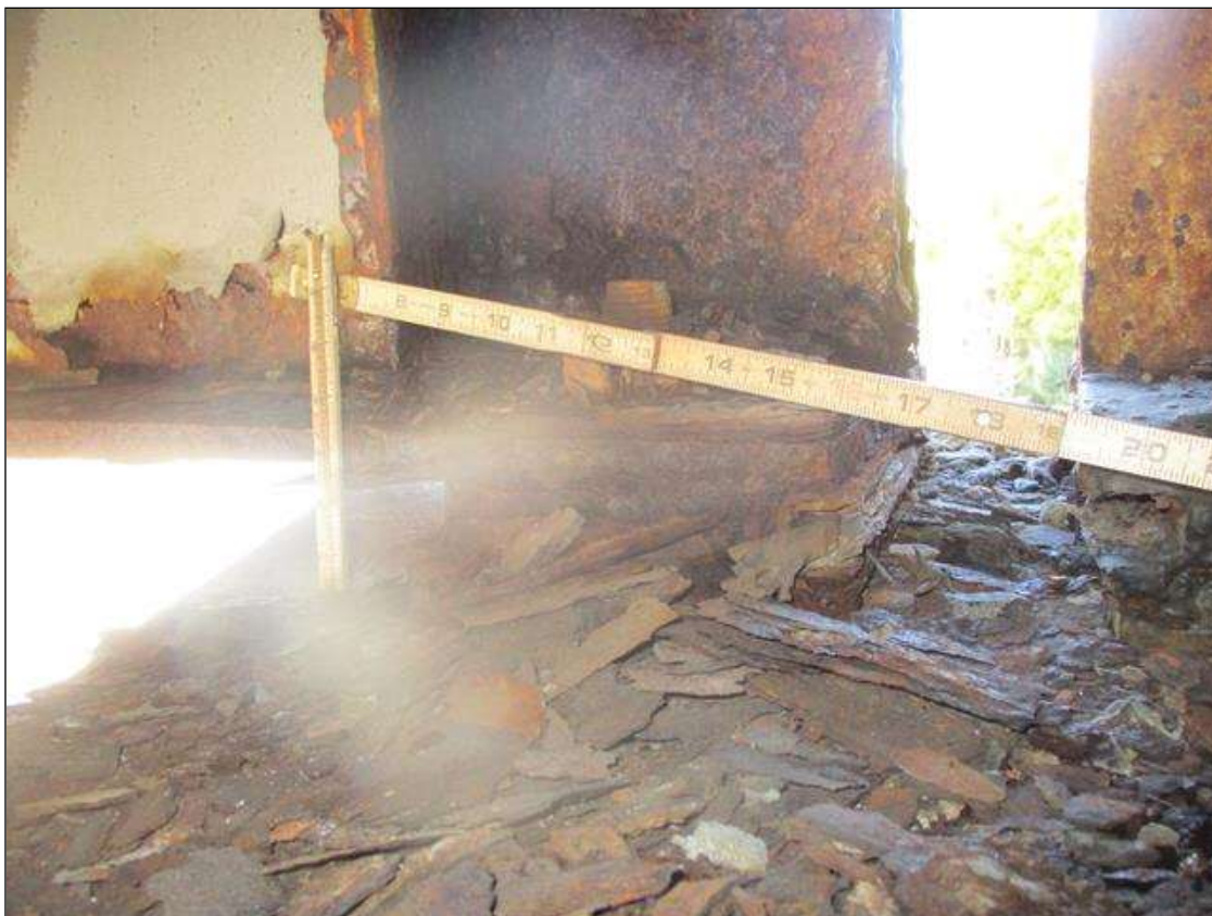
Span 3 Beam 1: BOTTOM FLANGE SECTION LOSS (UP TO 27%, 1/4IN SL, 11/16IN REMAIN) FULL WIDTH FOR 1FT L. AT FAR END. (PAR)
