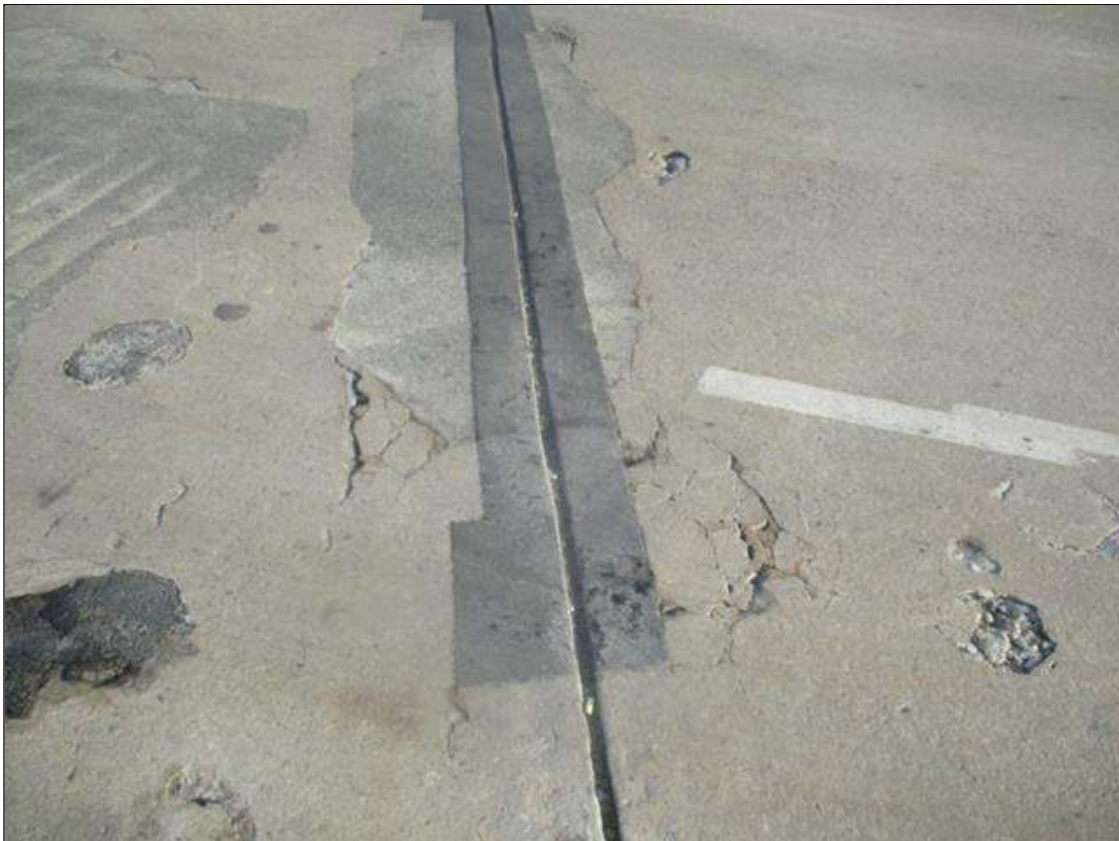
Span 2 Expansion Joint 2: PATCHING, (UP TO 2FT L. X FULL WIDTH) THROUGHOUT HEADERS
