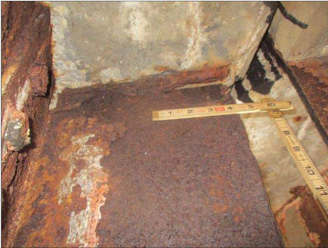
Span 4 Beam 8: WEB SECTION LOSS (UP TO 100%, AVG. 1/8IN REMAIN) TO TOP, 4IN L. X 1IN H.) AT NEAR END WITH REPAIR PLATE (3/4IN) AT RIGHT SIDE, PLATE DOES NOT COVER FULL HT. OF WEB (PAR)
