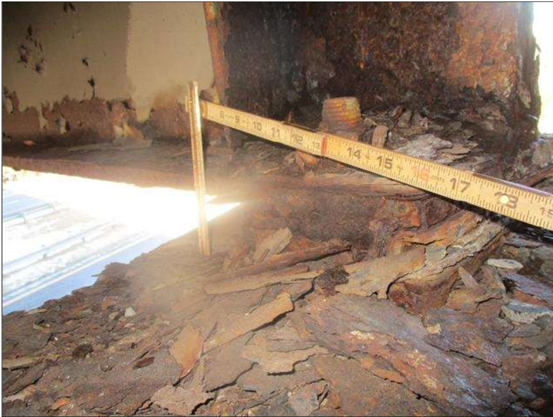
Span 3 Beam 1: BOTTOM FLANGE SECTION LOSS (UP TO 47%, 7/16IN SL, 1/2IN REMAIN) FULL WIDTH FOR 1FT L. AT NEAR END WITH REPAIR PLATES (3/4IN) TO WEB (FULL HT X 2FT L.) & STIFFENER (FULL HT. X FULL WIDTH). (PAR)
