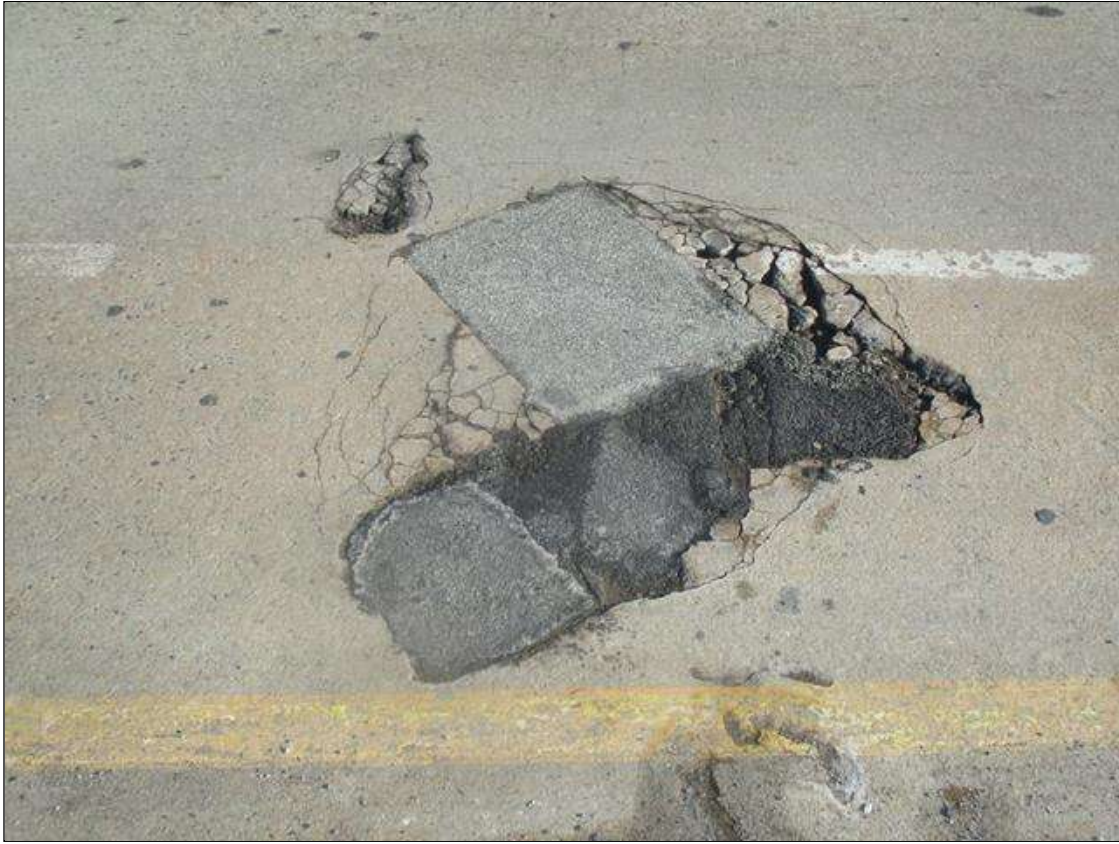
Span 3 Deck: SPALL WITH EXPOSED REBAR UP TO 12 SQ FT IN NORTHBOUND LAND RIGHT SIDE NEAR YELLOW LINE 20 FT FROM BENT 3. UP TO 90% SECTION REMAINING IN THE EXPOSED REBAR. (PAR)
