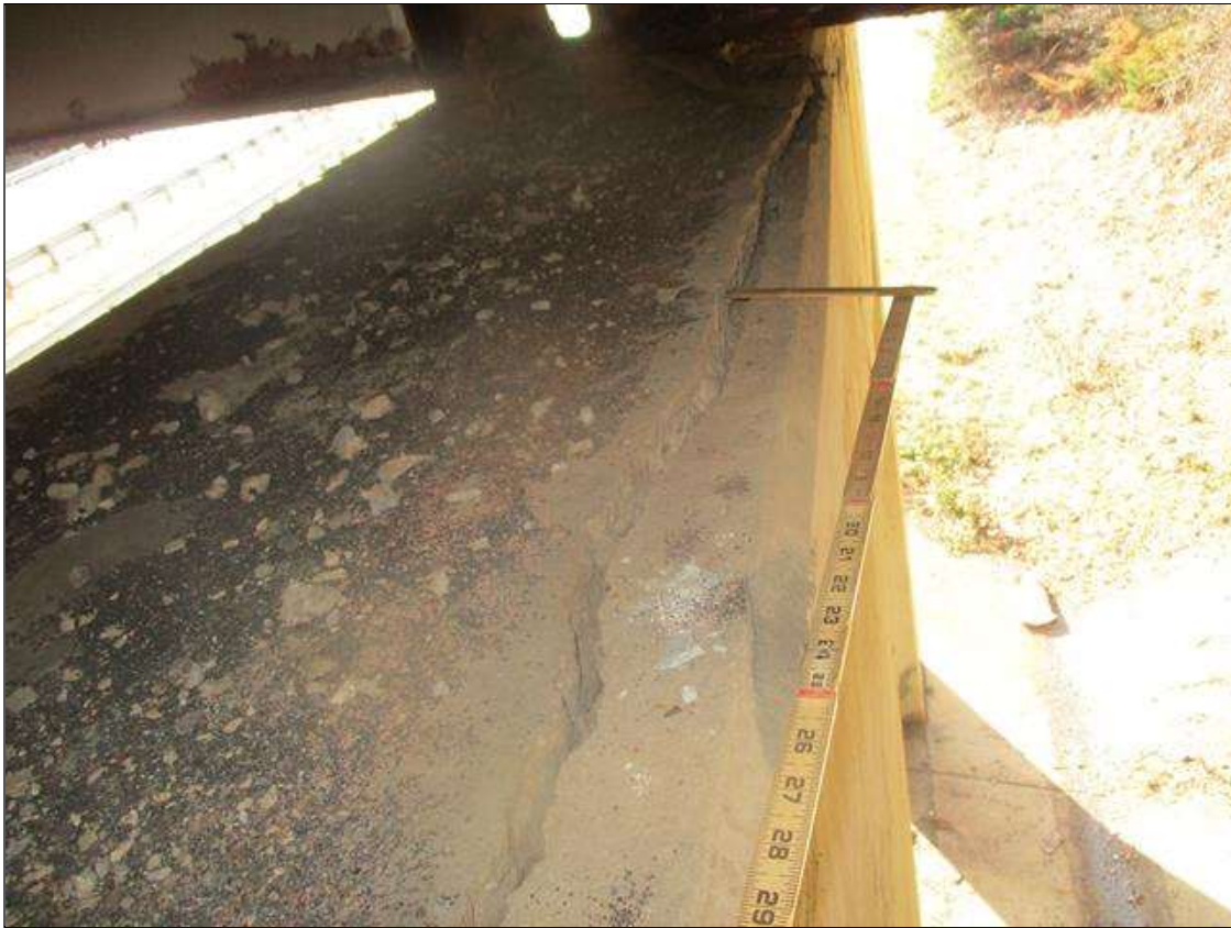
Bent 1 Cap 1: SPALL (2FT L. X 1FT H. X 8IN D.) WITH EXPOSED REINFORCING WITH UP TO 80% SECTION REMAINING IN THE EXPOSED REBAR AT THE BOTTOM EDGE TO THE LEFT OF COLUMN 4, NEAR FACE UNDER BEAM 7 & DELAM (16SF) WITH CRACK UP TO ONE IN WIDE TO TOP & BOTTOM EDGE (DELAM NOT UNDER BEARING) WITH RUST STAINING, NEAR FACE AT BAY 8, FAR FACE SIMILAR & DELAM (16SF) TO TOP & BOTTOM EDGE (DELAM NOT UNDER BEARING) WITH RUST STAINING, FAR FACE AT BAY 6 & DELAM (12SF) TO TOP EDGE (DELAM NOT UNDER BEARING), FAR FACE OVER COLUMN 1
