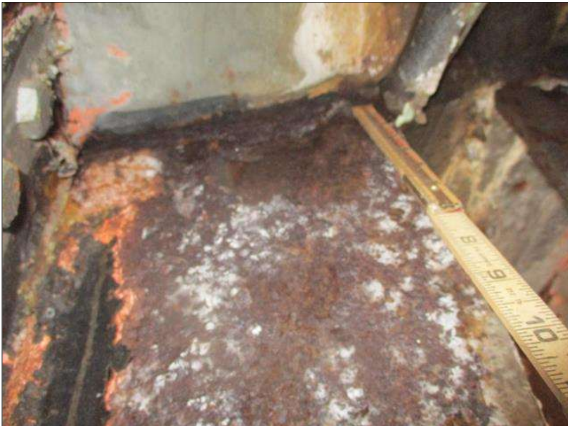
Span 4 Beam 7: WEB SECTION LOSS (UP TO 1/4IN SL, AVG. 3/8IN REMAIN) TO TOP, 5IN H. FOR 8IN L. AT NEAR END. (PAR)
