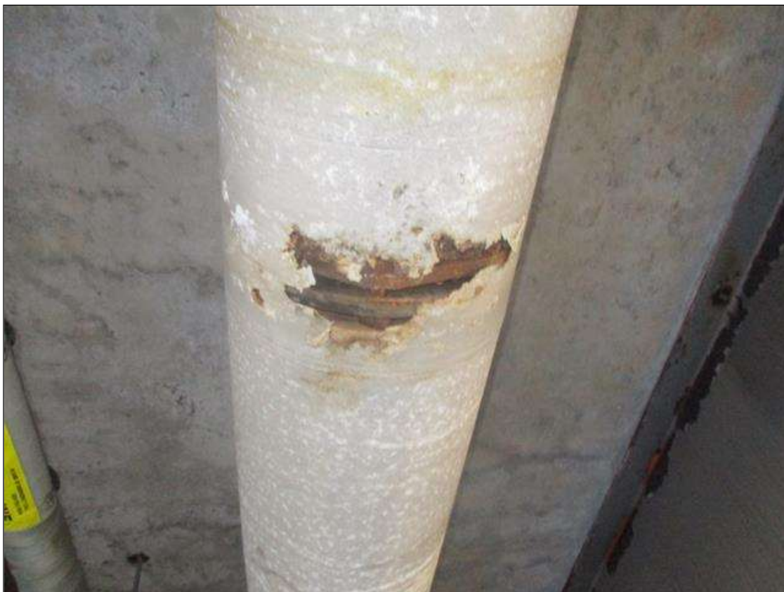
15 IN DIAMETER ULITLITY I BAY 1 HAS UP TO 100% CROSION APPROX. 15 FT FROM END BENT 2. SIMILAR AT END BENT 2.
