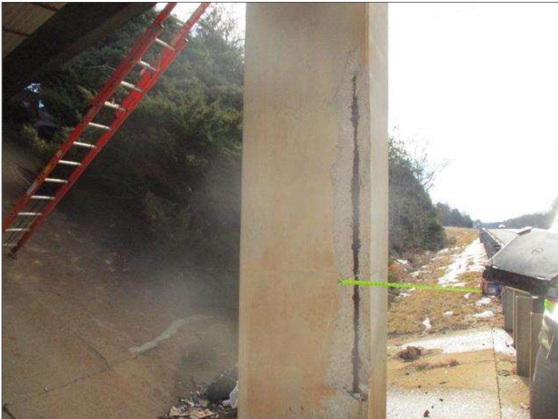
Bent 3 Pile 5: SPALL (7.5FT H. X 12N WIDE X 3IN D.) WITH EXPOSED REINFORCING, TO NEAR LEFT CORNER AT BOTTOM. UP TO 90% SECTION REMAINING IN THE EXPOSED REBAR. (PAR)
