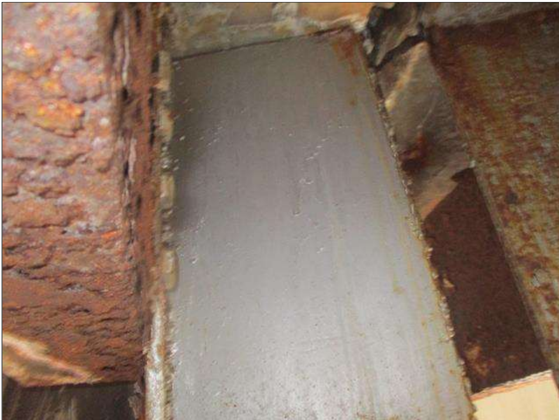
Span 4 Beam 9: WEB SECTION LOSS (UP TO 100%, AVG. 1/8IN REMAIN) TO TOP, 4IN L. FOR 2IN H. AT NEAR END WITH REPAIR PLATE (3/4IN X FULL HT.) AT LEFT SIDE. A REPAIR PLATE HAS BEEN INSTALLED.
