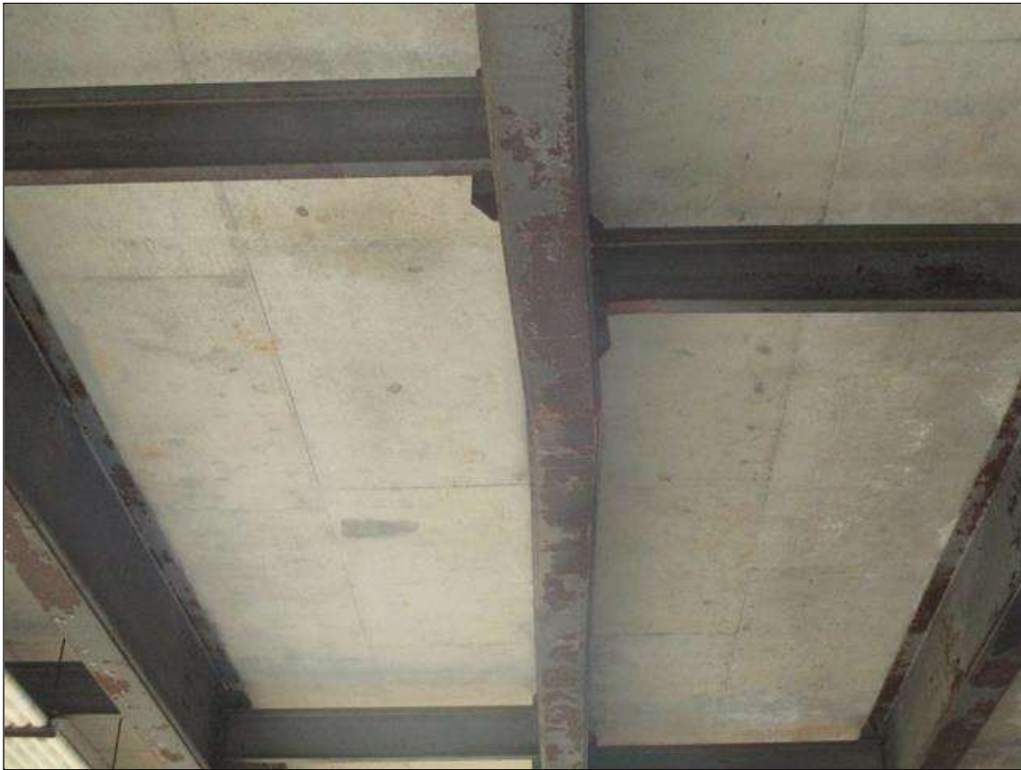
Span 3 Beam 8: IMPACT DAMAGE: 18"L SECTION OF BOTTOM FLANGE BENT UPWARD UP TO 2-1/2" AT 25' FROM BENT 3 BEARING. (PAR)
