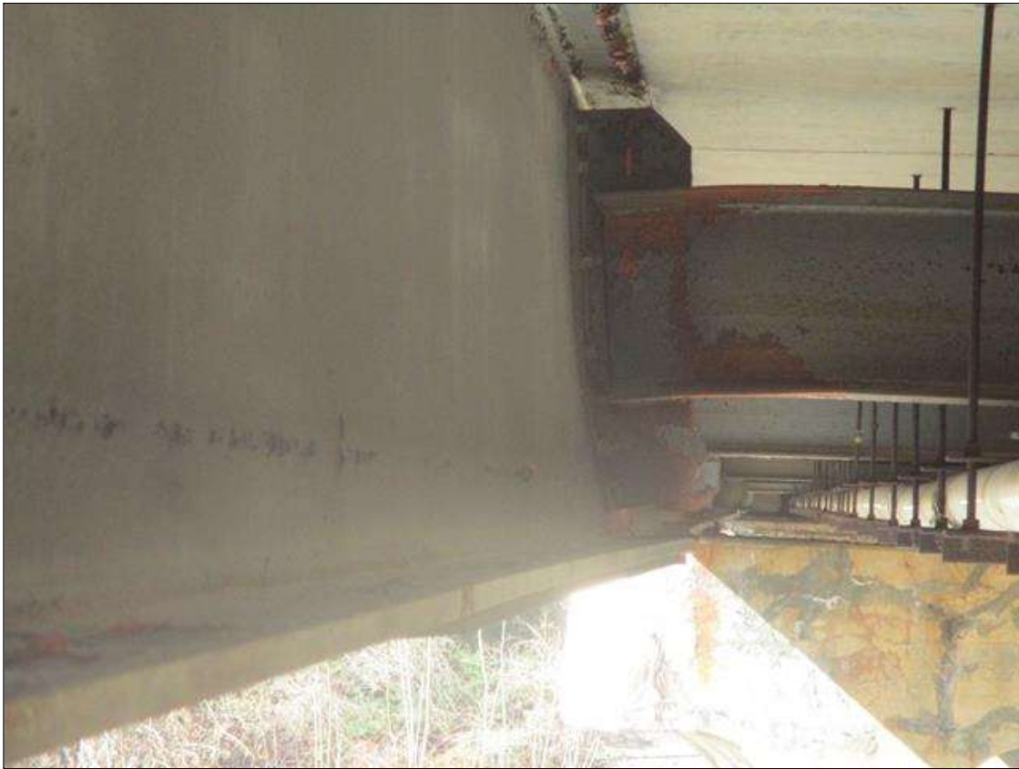
Span 3 Beam 10: IMPACT DAMAGE: 18" L SECTION OF BOTTOM FLANGE AND COVER PLATE BENT UPWARD UP TO 2-1/4" AT 24' FROM BENT 3 BEARING. (PAR)
