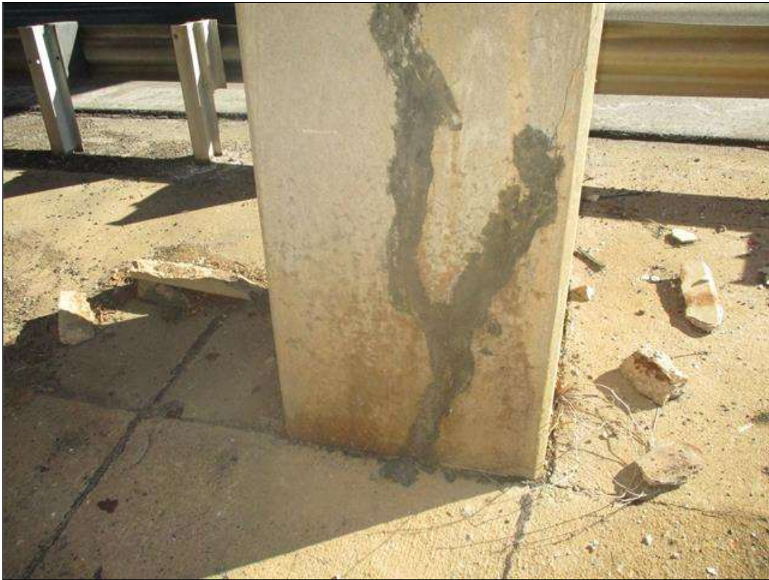
Bent 1 Pile 5: PARTIALLY SEALED CRACKS, (UP TO 1/32IN X FULL HT.) THROUGHOUT
