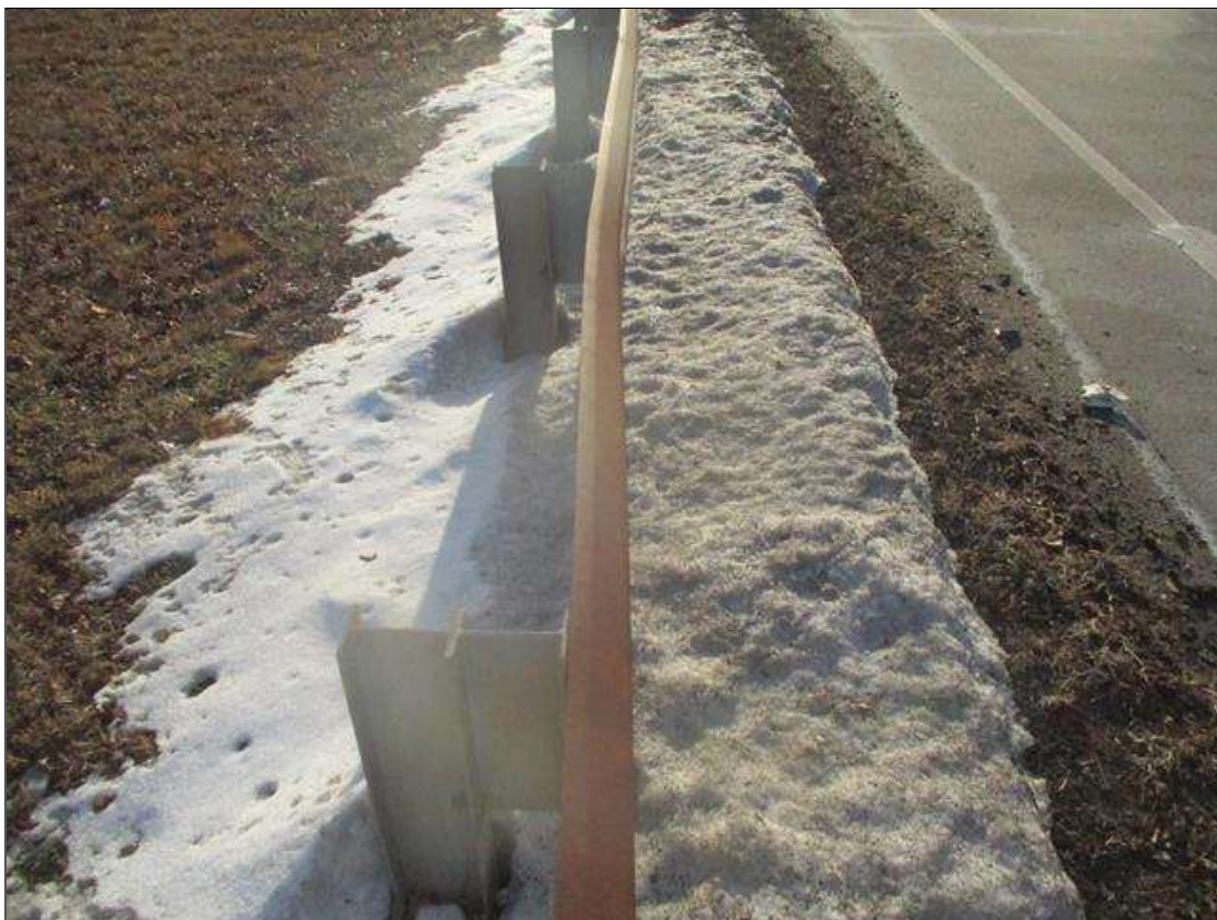
UP TO 6 FT OF IMPACT DAMAGE AT SOUTHEAST GUARDRAIL APPROX. 10 FT FROM BRIDGE
