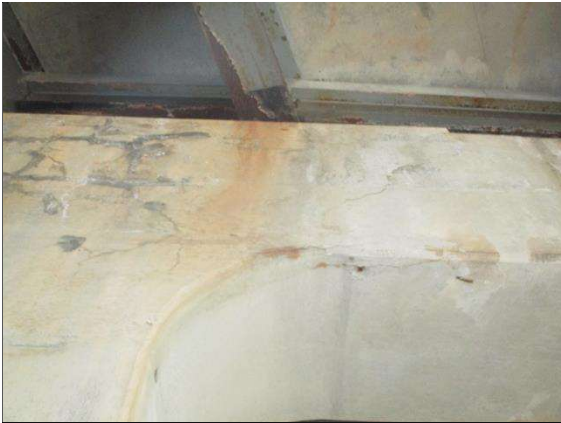
Bent 3 Cap 1: DELAM (14SF) TO BOTTOM EDGE, NEAR FACE AT BAY 2, SIMILAR AT FAR FACE & DELAM ( 8SF) TO NEAR FACE BELOW BEAM 6 (DEALM NOT UNDER BEARING) & DELAM ( 8SF) TO NEAR FACE BELOW BEAM 8 (DEALM NOT UNDER BEARING) & DELAM (8SF) TO BOTTOM EDGE, NEAR FACE UNDER BEAM 9. & DELAM (8SF) TO BOTTOM EDGE, FAR FACE BELOW BEAM 3
