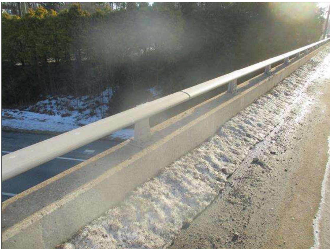
TYPICAL BRIDGE RAIL IN ALL SPANS BOTH SIDES. BOTTOM COVERED BY SNOW FOR FULL LENGTH IN BOTH SHOULDERS
