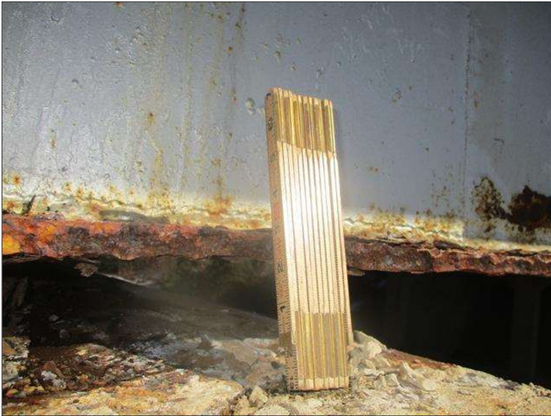
Span 3 Beam 10: BOTTOM FLANGE SECTION LOSS (UP TO 27%, 1/4IN SL, 11/16IN REMAIN) FULL WIDTH FOR 12IN L. AT NEAR END RIGHT SIDE (PAR).
