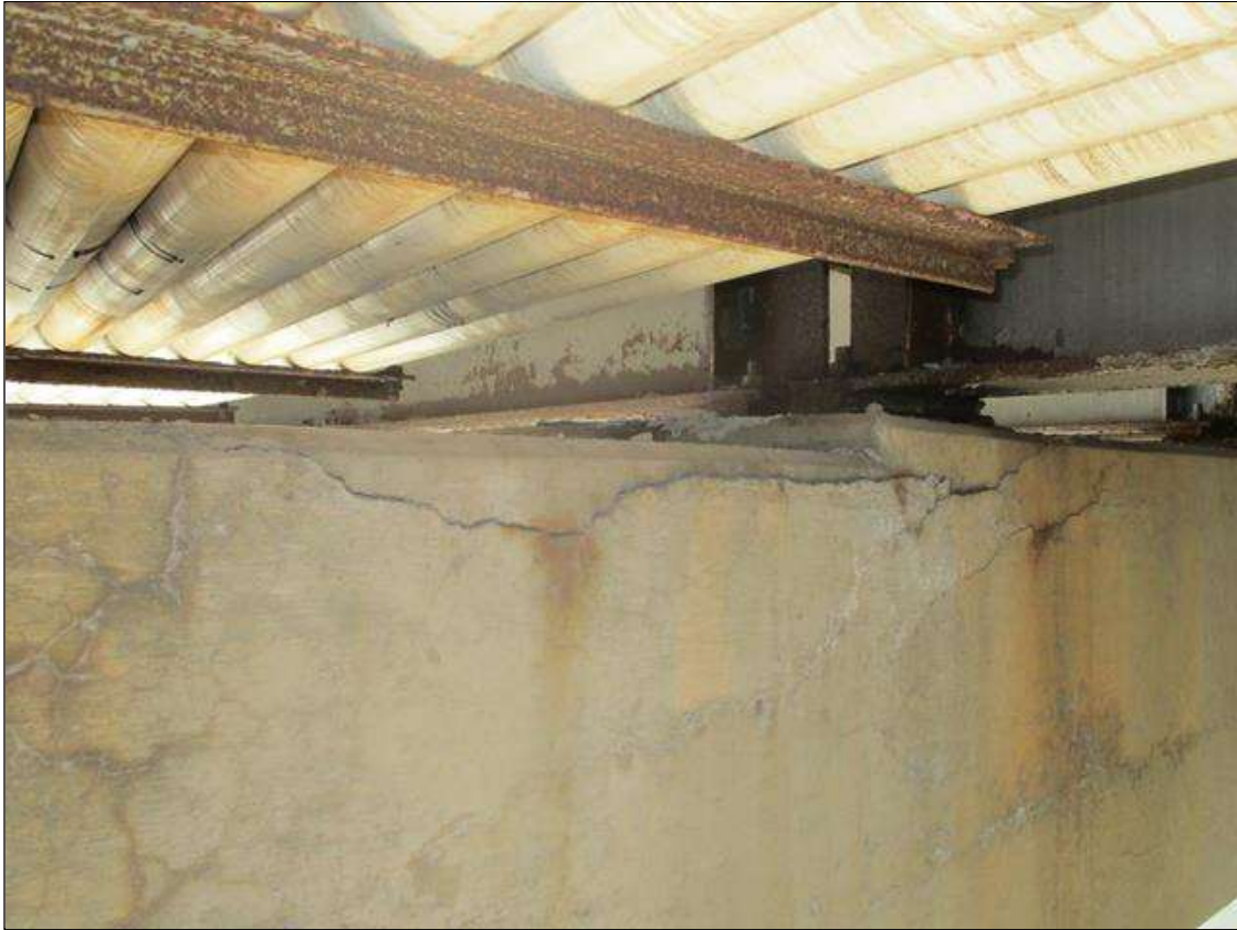
Bent 3 Cap 1: DELAM (14SF) TO BOTTOM EDGE, NEAR FACE AT BAY 2, SIMILAR AT FAR FACE & DELAM ( 8SF) TO NEAR FACE BELOW BEAM 6 (DEALM NOT UNDER BEARING) & DELAM ( 8SF) TO NEAR FACE BELOW BEAM 8 (DEALM NOT UNDER BEARING) & DELAM (8SF) TO BOTTOM EDGE, NEAR FACE UNDER BEAM 9. & DELAM (8SF) TO BOTTOM EDGE, FAR FACE BELOW BEAM 3
