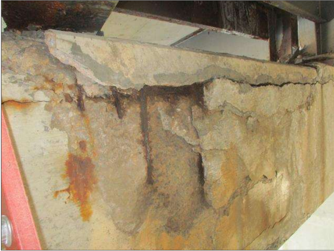
Bent 1 Cap 1: DELAM (16SF) TO TOP & BOTTOM EDGE (DELAM NOT UNDER BEARING), NEAR FACE AT BAY 4, FAR FACE SIMILAR & DELAM (5SF) NEAR FACE ABOVE COLUMN 3 & DELAM (16SF) TO TOP & BOTTOM EDGE (DELAM NOT UNDER BEARING). UP TO 80% SECTION REMAINING ON THE EXPOSED REBAR. SPALL UNDER BAY 4 IS UP TO 4 SQ FT. (PAR)
