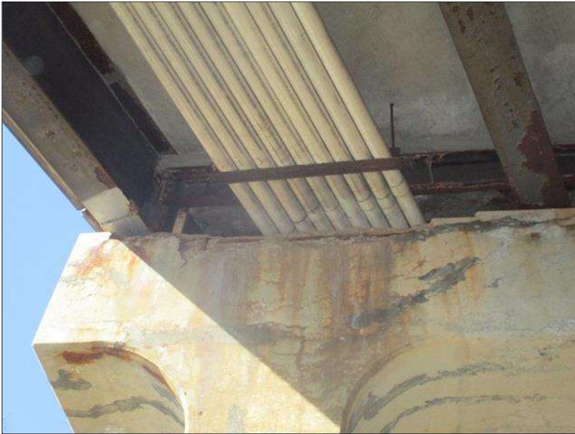
Bent 1 Cap 1: SPALL (7FT L. X 1FT WEST. X 4IN D.) WITH EXPOSED REINFORCING TO TOP EDGE, FAR FACE AT BAY 9. UP TO 90% SECTION REMAINING IN THE EXPOSED REBAR. (PAR) - COULD NOT ACCESS WITH LADDER DUE TO PROXIMITY OF LIVE TRAFFIC AT FAR FACE OF BENT.
