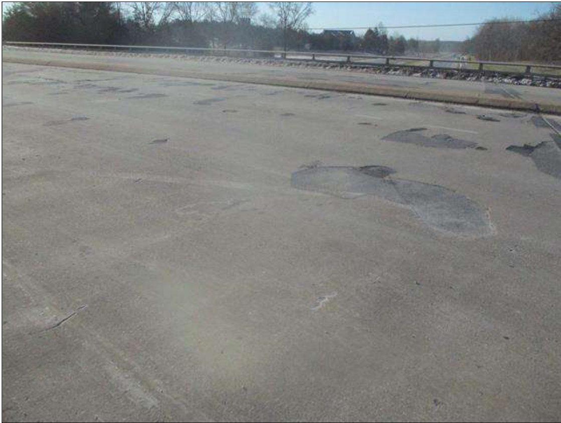
TOP OF DECK - WITH PATCHED SPALLS SCATTERED THROUGHOUT
