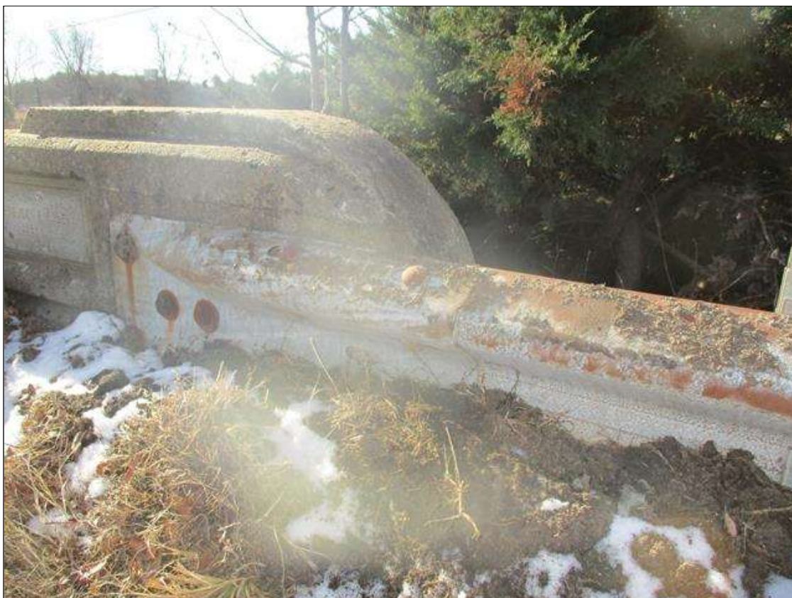
APPROACH GUARDRAIL AT NORTHWEST CORNER IS LAPPED INCORRECTLY (PAR)
