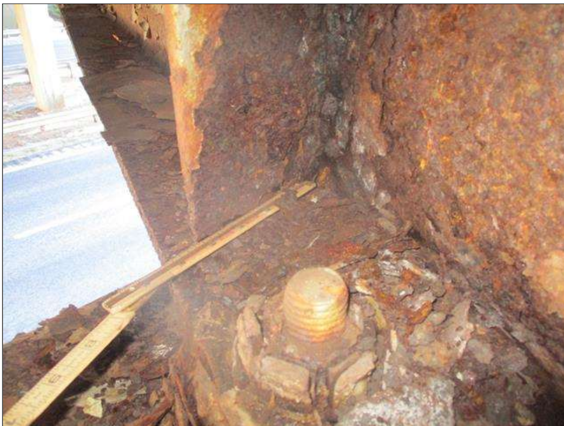
Span 3 Beam 1: FAR END, RIGHT STIFFENER SECTION LOSS (UP TO 100%) FOR 4 IN WIDE AT BOTTOM. (PAR)
