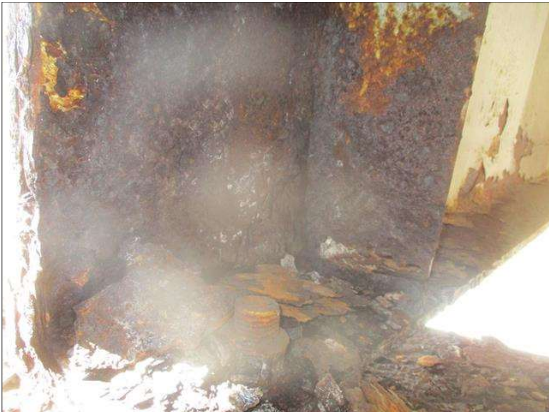
Span 3 Beam 10: LEFT STIFFENER SECTION LOSS (UP TO 100%) TO BOTTOM FOR FULL WIDTH X 1 IN HIGH. (PAR)
