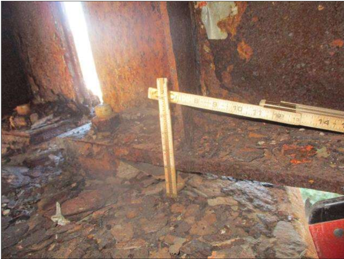
Span 4 Beam 1: BOTTOM FLANGE SECTION LOSS (UP TO 27%, 1/4IN SL, 11/16IN REMAIN) FULL WIDTH FOR 2FT L. AT NEAR END & RIGHT STIFFENER SECTION LOSS (AVG. 1/4IN REMAIN) TO BOTTOM 3IN. (PAR)
