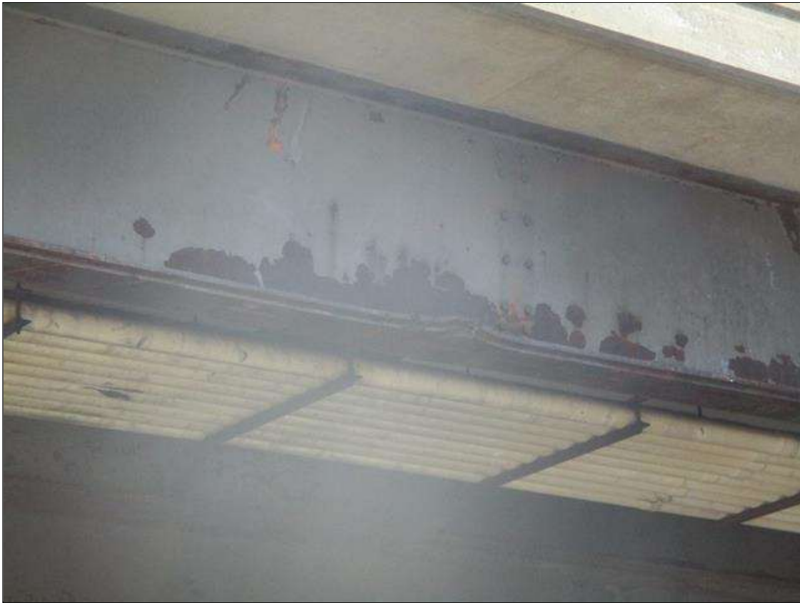
Span 3 Beam 10: IMPACT DAMAGE: 18"L SECTION OF BOTTOM FLANGE AND COVER PLATE BENT UPWARD UP TO 2-1/4" AT 24' FROM BENT 3 BEARING. (PAR)
