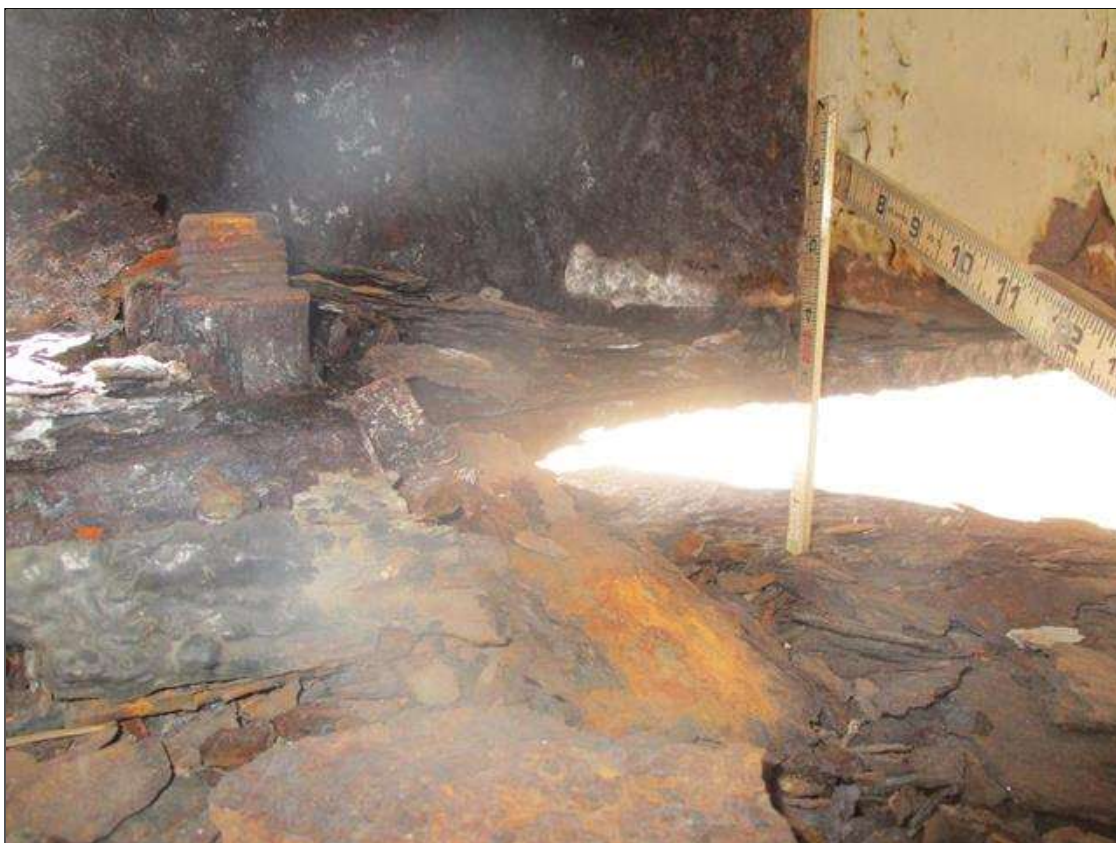
Span 3 Beam 10: BOTTOM FLANGE SECTION LOSS (UP TO 53%, 1/2IN SL, 7/16IN REMAIN) FULL WIDTH FOR 1FT L. AT FAR END. (PAR)
