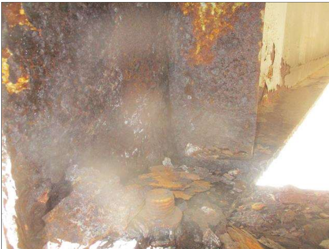
Span 3 Beam 10: LEFT STIFFENER SECTION LOSS (UP TO 100%) TO BOTTOM FOR FULL WIDTH X 1 IN HIGH. (PAR)
