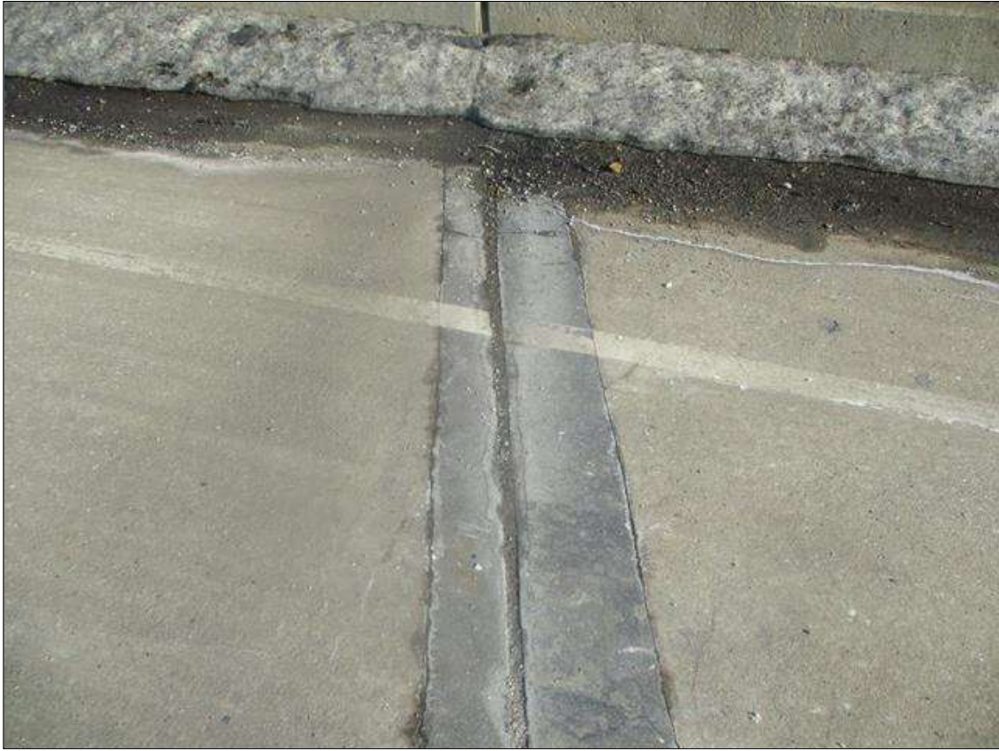
Span 2 Expansion Joint 2: DEBRIS IMPACTION FULL L.
