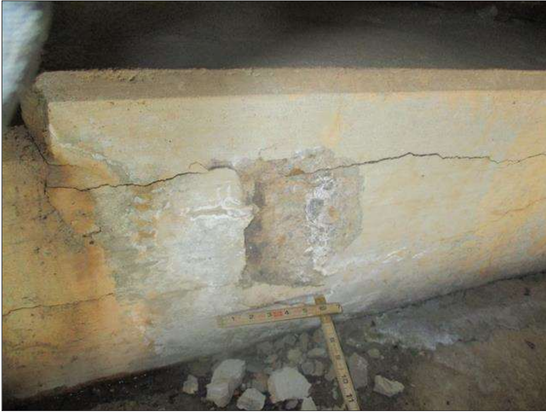
End Bent 2 Cap 1: SPALL (8IN X 8IN X 1.5IN) WITH EXPOSED REINFORCING (UP TO 90% SECTION REMAINING IN THE EXPOSED REBAR), FAR FACE AT BEAM 3 & SPALLING/DELAM (5FT L. X 6IN WIDE X 2IN D.) NO EXPOSED REINFORCING, FAR FACE TOP EDGE AT RIGHT END
