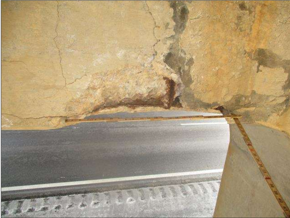
Bent 1 Cap 1: SPALL (2FT L. X 1FT H. X 8IN D.) WITH EXPOSED REINFORCING WITH UP TO 80% SECTION REMAINING IN THE EXPOSED REBAR AT THE BOTTOM EDGE TO THE LEFT OF COLUMN 4, NEAR FACE UNDER BEAM 7 & DELAM (16SF) WITH CRACK UP TO ONE IN WIDE TO TOP & BOTTOM EDGE (DELAM NOT UNDER BEARING) WITH RUST STAINING, NEAR FACE AT BAY 8, FAR FACE SIMILAR & DELAM (16SF) TO TOP & BOTTOM EDGE (DELAM NOT UNDER BEARING) WITH RUST STAINING, FAR FACE AT BAY 6 & DELAM (12SF) TO TOP EDGE (DELAM NOT UNDER BEARING), FAR FACE OVER COLUMN 1
