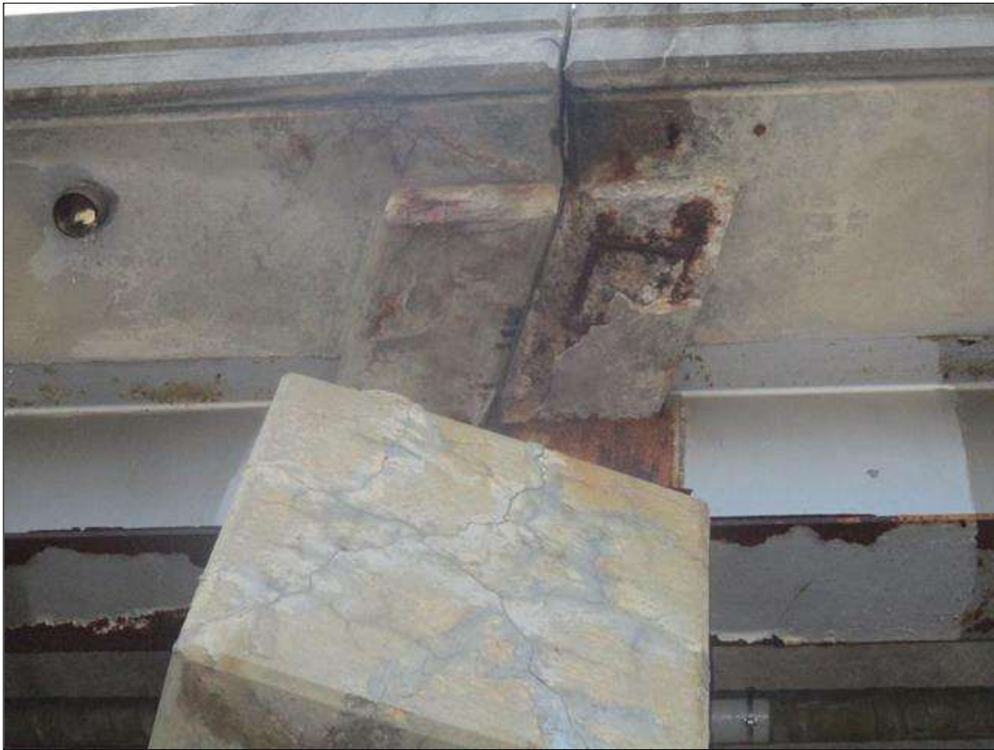
Span 2 Deck: UNDERSIDE OF DECK, LEFT OVERHANG - SPALL (18IN X 12IN X 3IN) WITH EXPOSED REINFORCING, FAR END. UP TO 80% SECTION REMAINING IN THE EXPOSED REBAR (PAR)
