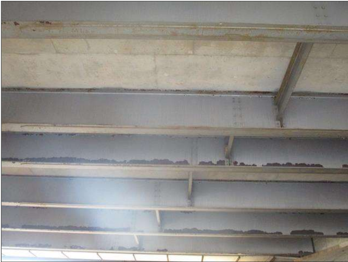
Span 1 Beam 6 - Protective System: PC LOSS AT CORRODED AREAS & PEELING THROUGHOUT FLANGES & BOTTOM 1/3 OF WEB
