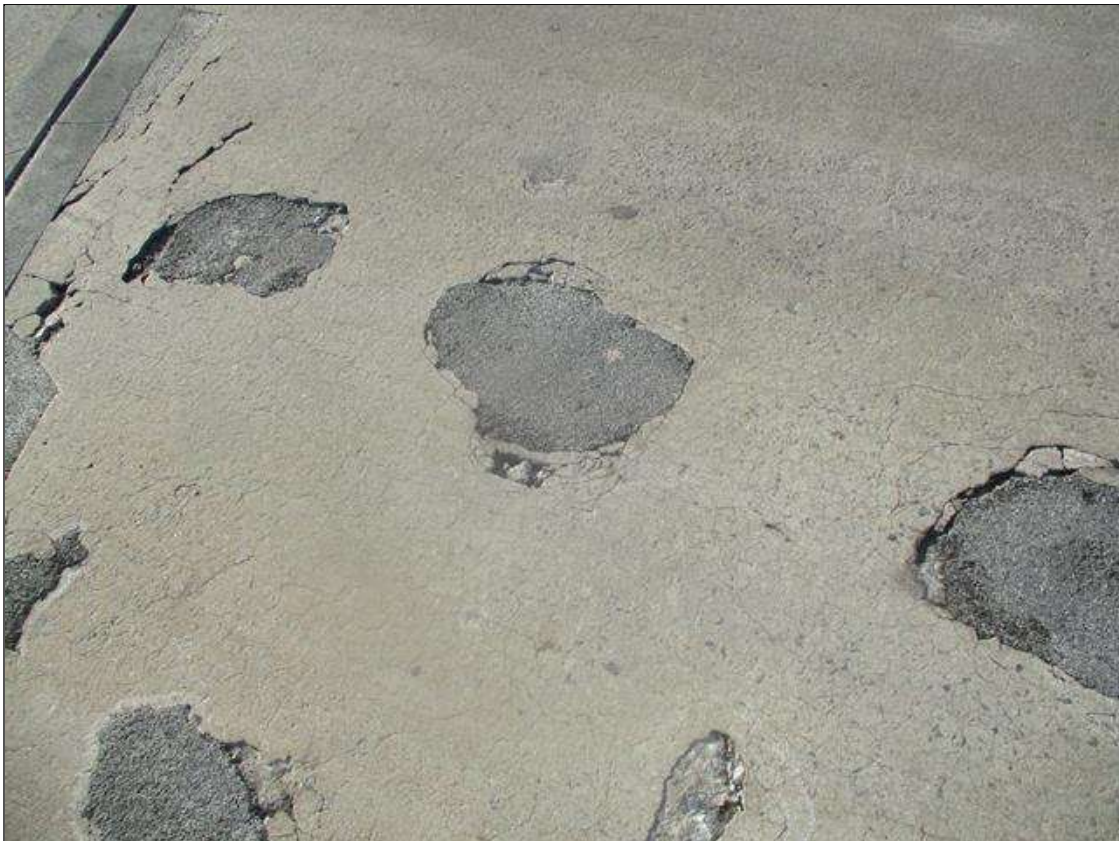
Span 3 Deck: SPALL (16IN X 12IN X 2IN) WITH EXPOSED REINFORCING, RIGHT LANE 3FT FROM FAR END. PATCHED SINCE PREVIOUS INSPECTION - NEW REPAIR
