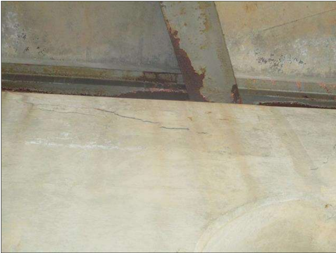
Bent 3 Cap 1: DELAM (14SF) TO BOTTOM EDGE, NEAR FACE AT BAY 2, SIMILAR AT FAR FACE & DELAM ( 8SF) TO NEAR FACE BELOW BEAM 6 (DEALM NOT UNDER BEARING) & DELAM ( 8SF) TO NEAR FACE BELOW BEAM 8 (DEALM NOT UNDER BEARING) & DELAM (8SF) TO BOTTOM EDGE, NEAR FACE UNDER BEAM 9. & DELAM (8SF) TO BOTTOM EDGE, FAR FACE BELOW BEAM 3
