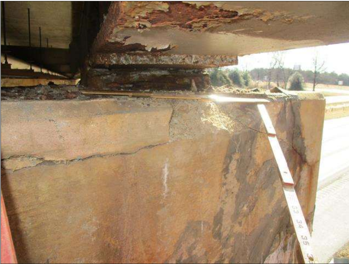
Bent 1 Cap 1: SPALL UP TO 18 IN LONG X 3 IN HIGH X 4 IN DEEP IN NEAR FACE BELOW BEAM 10. NO EXPOSED REBAR AND NOT UNDERMINING THE MASONRY PLATE
