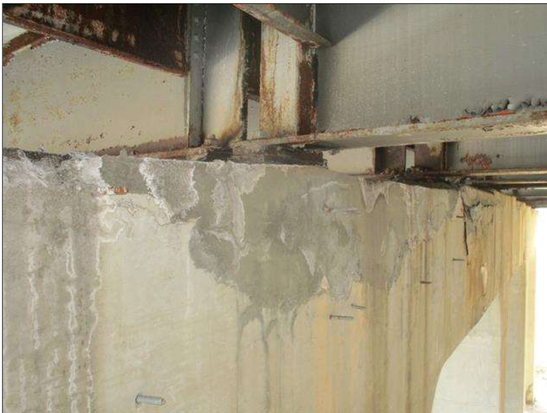
Bent 1 Cap 1: PATCH (10FT L. X FULL WIDTH AND UP TO 18 IN HIGH) WITH DELAM (3FT L. X FULL WIDTH) AT RIGHT END OF PATCH, NEAR FACE ABOVE COLUMN 2
