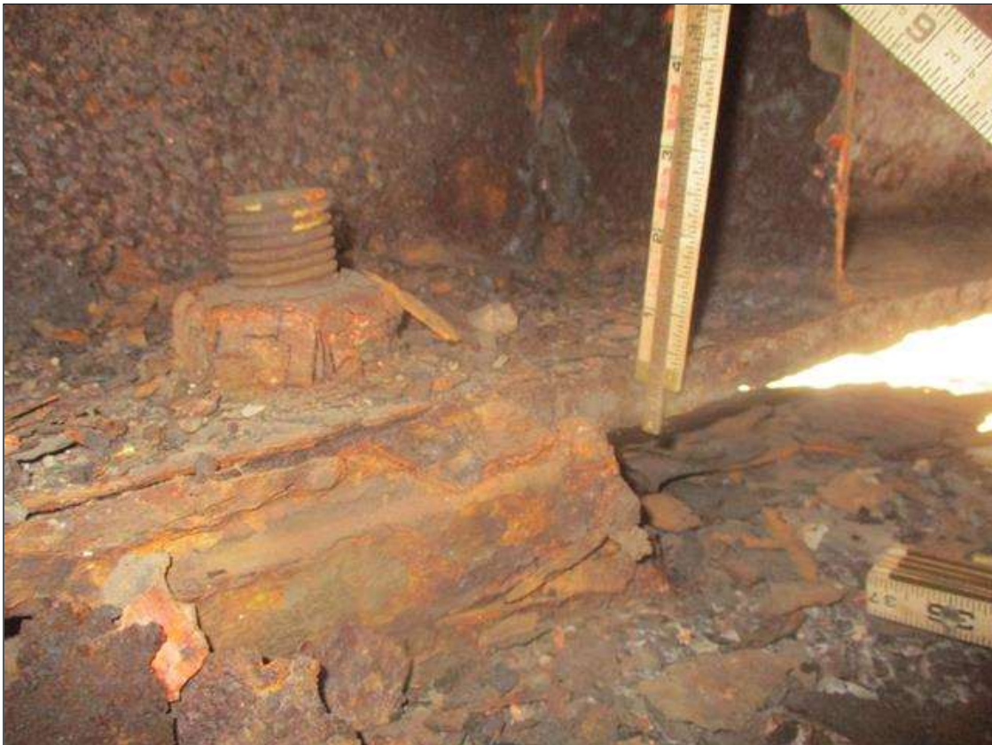
Span 3 Beam 6: BOTTOM FLANGE SECTION LOSS (UP TO 27%, 1/4IN SL, 11/16IN REMAIN) FULL WIDTH FOR 1FT L. AT FAR END & LEFT STIFFENER SECTION LOSS (AVG. 5/16IN REMAIN) TO BOTTOM 3IN. (PAR)
