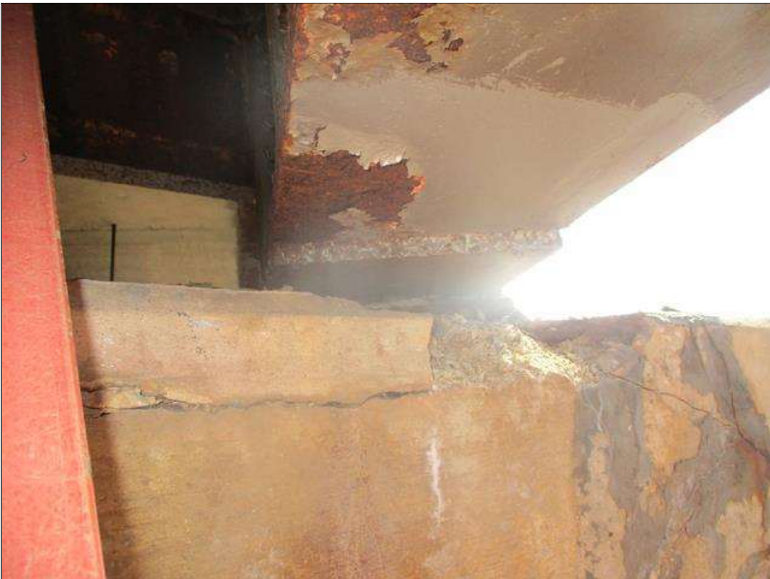
Span 1 Beam 10: REPAIR PLATE (3/4IN) TO BOTTOM FLANGE (8IN L. X FULL WIDTH) AT FAR END
