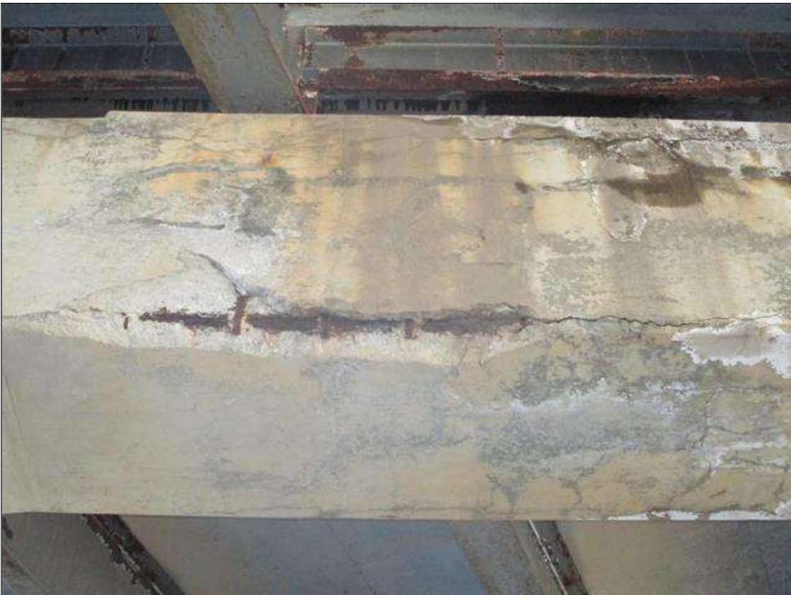
Bent 2 Cap 1: SPALLING/DELAM (10SF X 4IN D.) WITH EXPOSED REINFORCING TO BOTTOM EDGE, NEAR FACE AT BAY 4. UP TO 70% SECTION REMAINING IN THE EXPOSED REBAR. (PAR)
