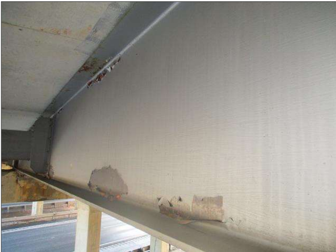
Span 1 Beam 4: MINOR SURFACE CORROSION THROUGHOUT FLANGES & BOTTOM 1/3 OF WEB
