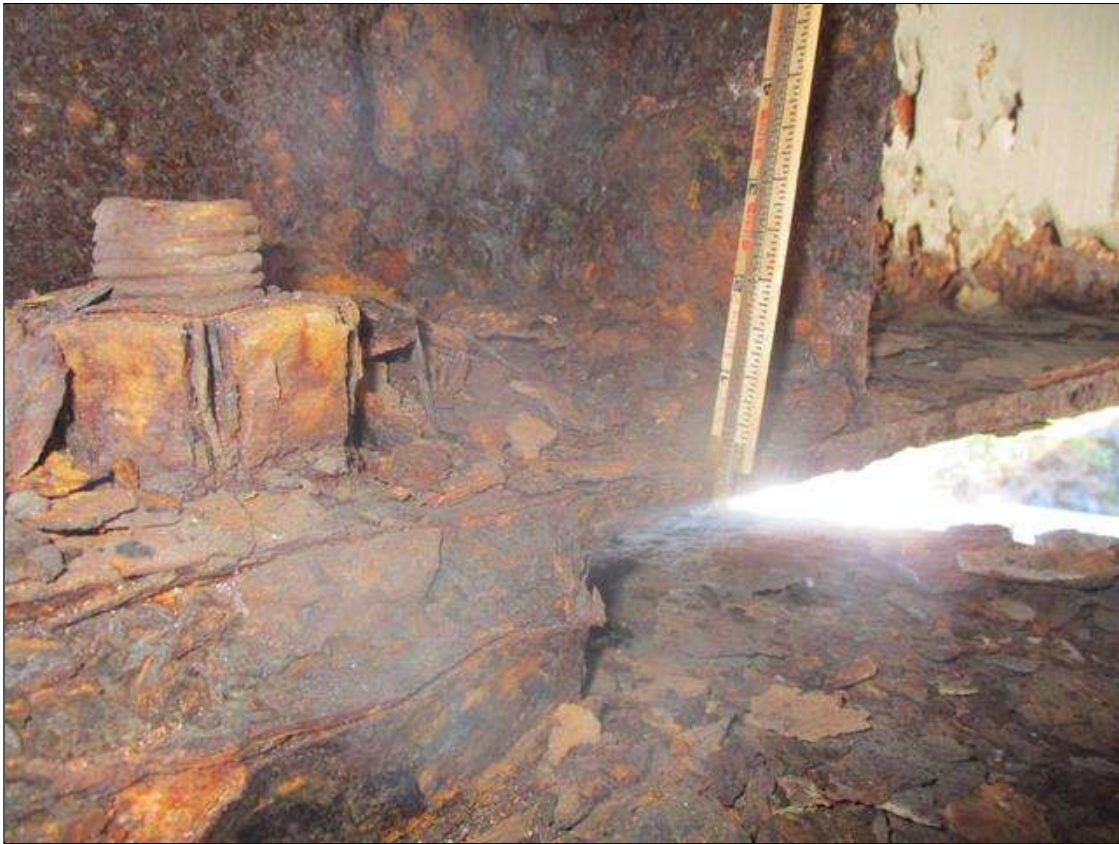
Span 3 Beam 1: BOTTOM FLANGE SECTION LOSS (UP TO 47%, 7/16IN SL, 1/2IN REMAIN) FULL WIDTH FOR 1FT L. AT NEAR END WITH REPAIR PLATES (3/4IN) TO WEB (FULL HT X 2FT L.) & STIFFENER (FULL HT. X FULL WIDTH). (PAR)
