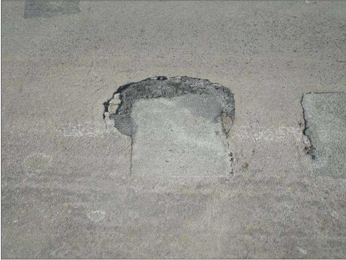
Span 2 Deck: SPALL (14IN X 12IN X 2IN) WITH EXPOSED REINFORCING, RIGHT LANE 16FT FROM FAR END. - PATCHED SINCE PREVIOUS INSPECTION, NEW REPAIR
