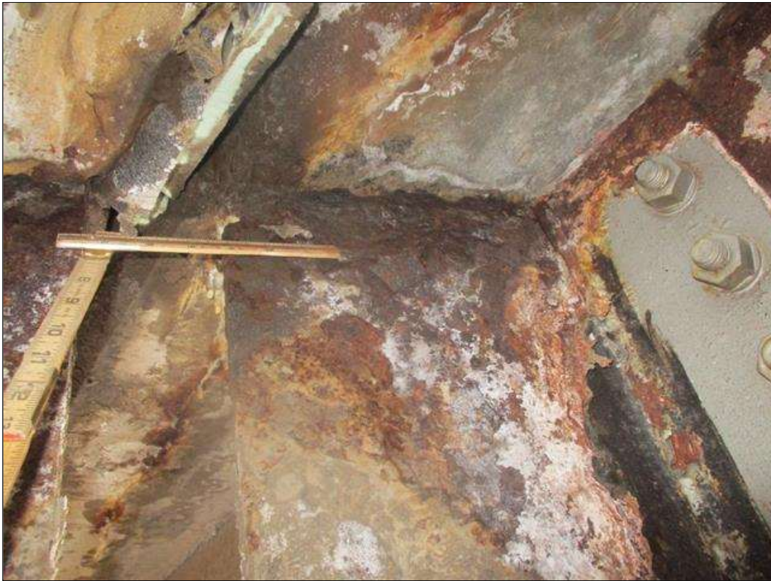
Span 3 Beam 7: WEB SECTION LOSS (UP TO 100%, AVG. 1/8IN REMAIN) TO TOP, 3IN L. FOR 1IN H. AT FAR END (PAR)
