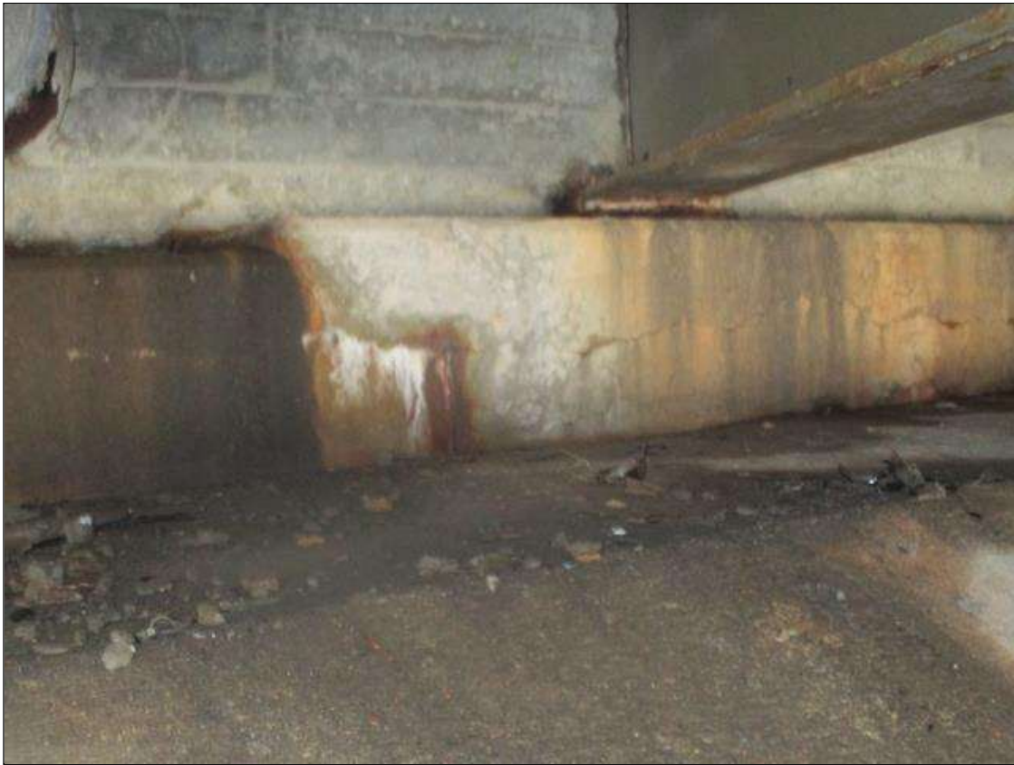
End Bent 2 Cap 1: HORIZONTAL 1/16IN CRACKING (UP TO FULL L.) WITH EFFLO. & RUST STAINING THROUGHOUT
