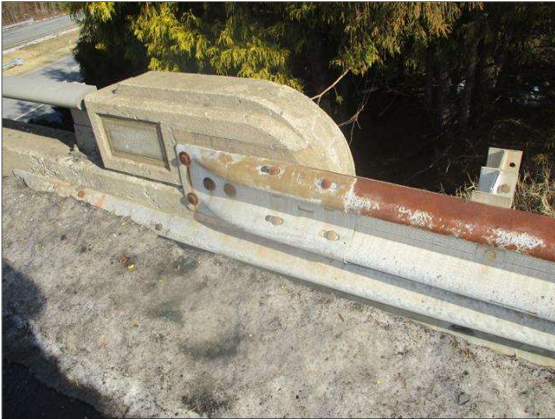
INCORRECT LAPPING AT SOUTHEAST GUARDRAIL TRANSITION (PAR)
