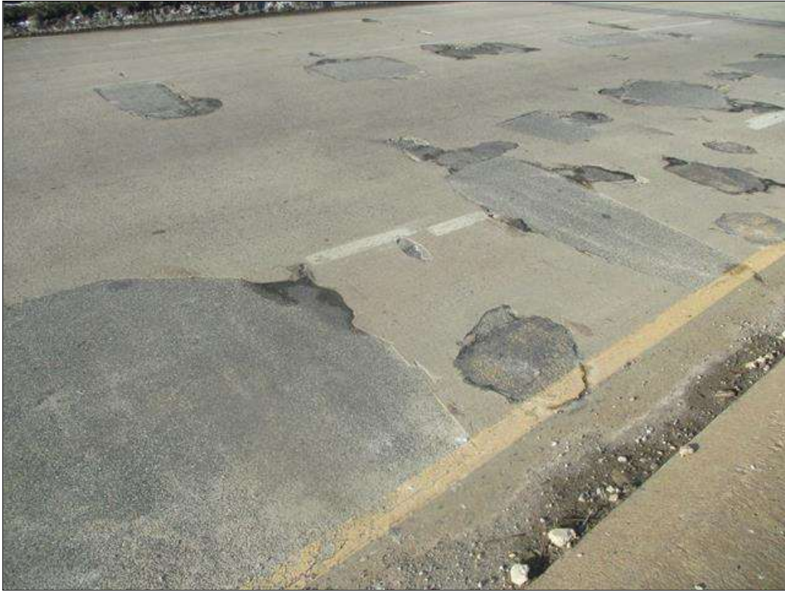
Span 2 Deck: INTERMITTENT PATCHING (UP TO 50SF) WITH SPALLING (UP TO 12IN X 12IN X 1IN) AT PERIMETER OF PATCHING
