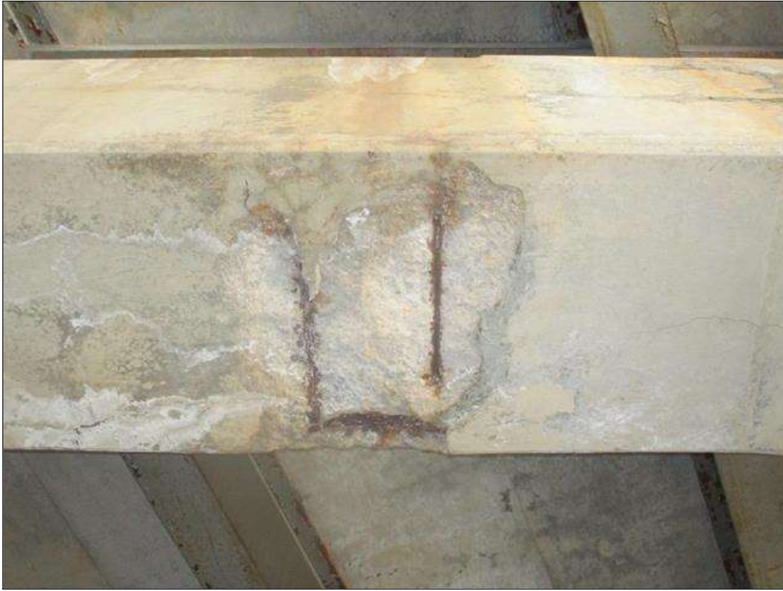
Bent 3 Cap 1: SPALL (10SF X 4IN D.) WITH EXPOSED REINFORCING, UNDERSIDE AT BAY 4. UP TO 80% SECTION REMAINING IN THE EXPOSED BAR. (PAR)
