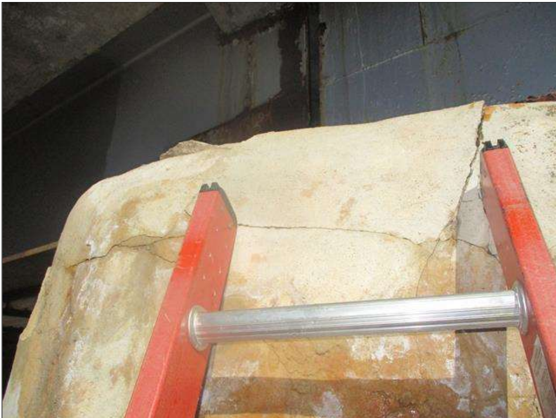
Bent 2 Cap 1: POOR PATCH (3SF) WITH OPEN 1/32IN MAP CRACKING WITH RUST STAINING & EFFLO. THROUGHOUT, RIGHT END
