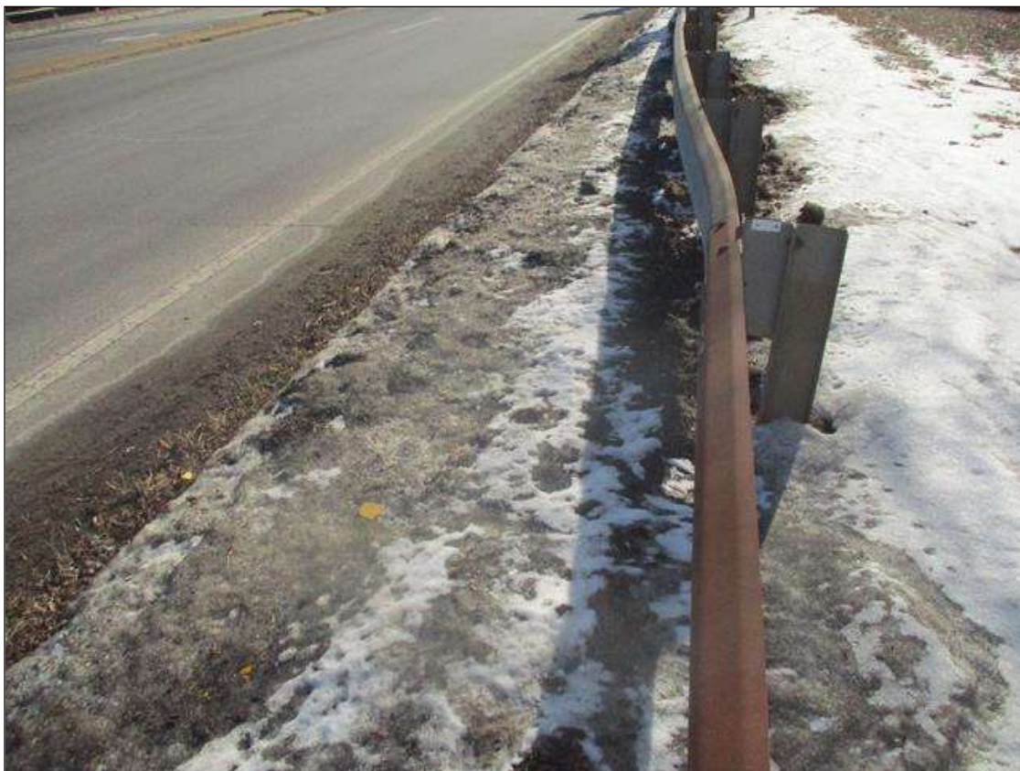
MODERATE IMPACT DAMAGE TO NORTHWEST GUARDRAIL APPROX. 50 FT FROM BRIDGE FOR 20 FT LONG.
