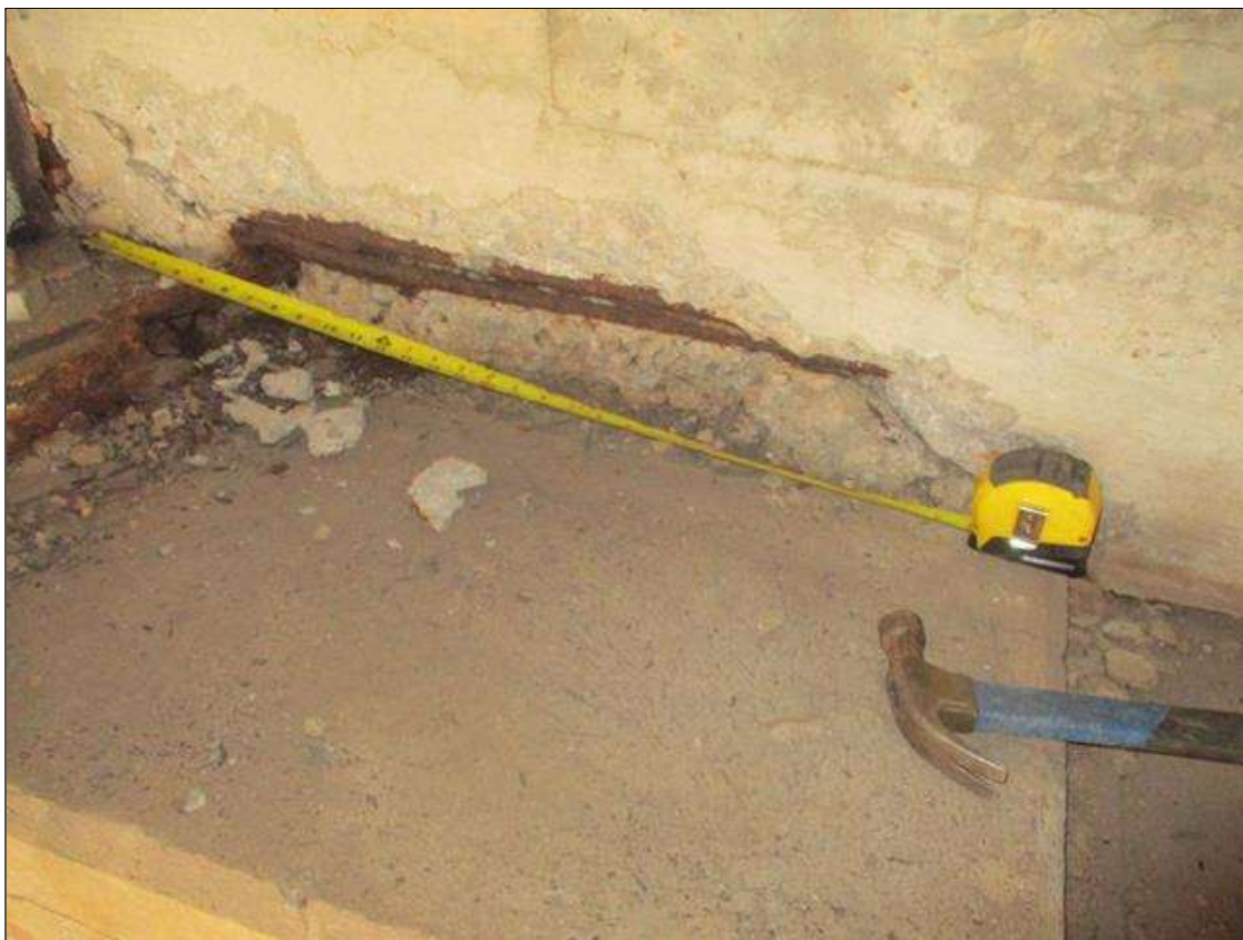
End Bent 2 Abutment: SPALL (30IN L. X 9IN H. X 3IN D.) WITH EXPOSED REINFORCING TO BOTTOM OF BACKWALL RIGHT OF BEAM 7. REBAR IS DEBONDED FOR FULL LENGTH OF SPALL AND HAS UP TO 90% SECTION REMAINING IN THE EXPOSED REBAR. (PAR)
