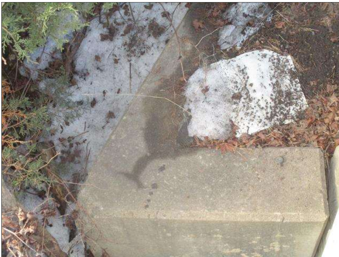
MINOR HAIRLINE MAP CRACKING AT SOUTHEAST WINGWALL.
