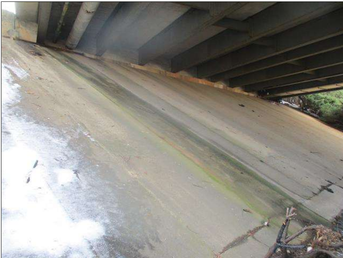
SLOPE PROTECTION AT END BENT 2
