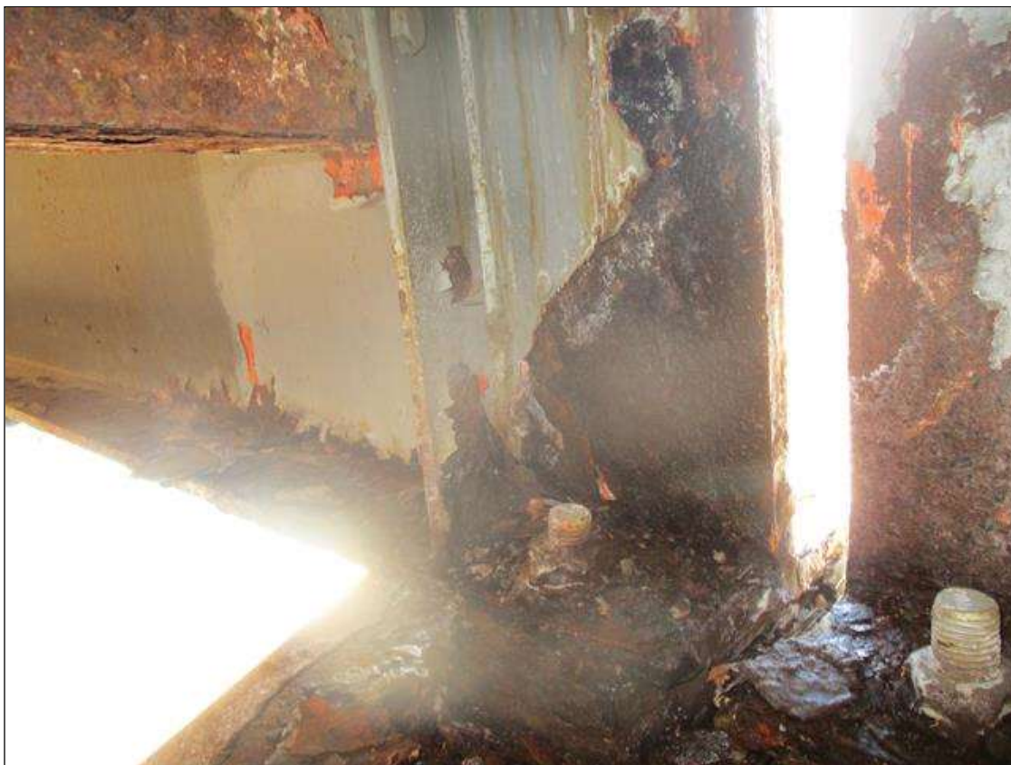
Span 3 Beam 10: REPAIR PLATES (3/4IN) TO WEB (3FT L. X 15IN H.) AT NEAR END
