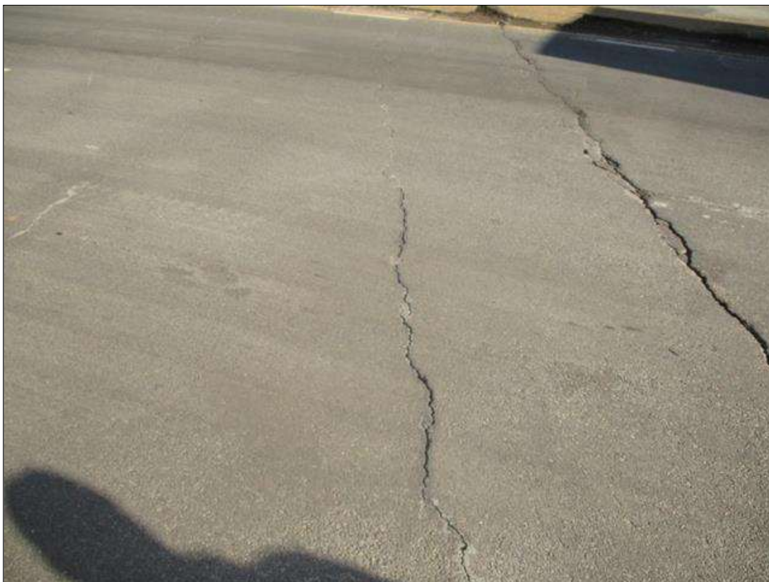
CRACKING UP TO 1/2 IN WIDE IN APPROACH PAVEMENT NEAR END BENT 1 FOR FULL WIDTH
