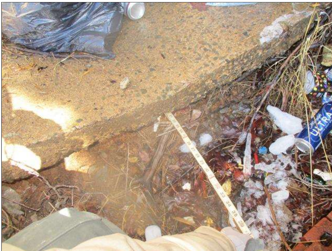
THERE IS EROSION BELOW THE CONCRETE APRON AT THE RIGHT END OF BENT 3 RESULTING IN A 5.5 FT LONG X 1 FT HIGH GAP WHICH CAN BE PROBED UP TO 21 IN DEEP. THIS IS THE RESULT OF A DISCONTINUITY IN THE APRON TO MAKE ROOM FOR A CATCH BASIN.
