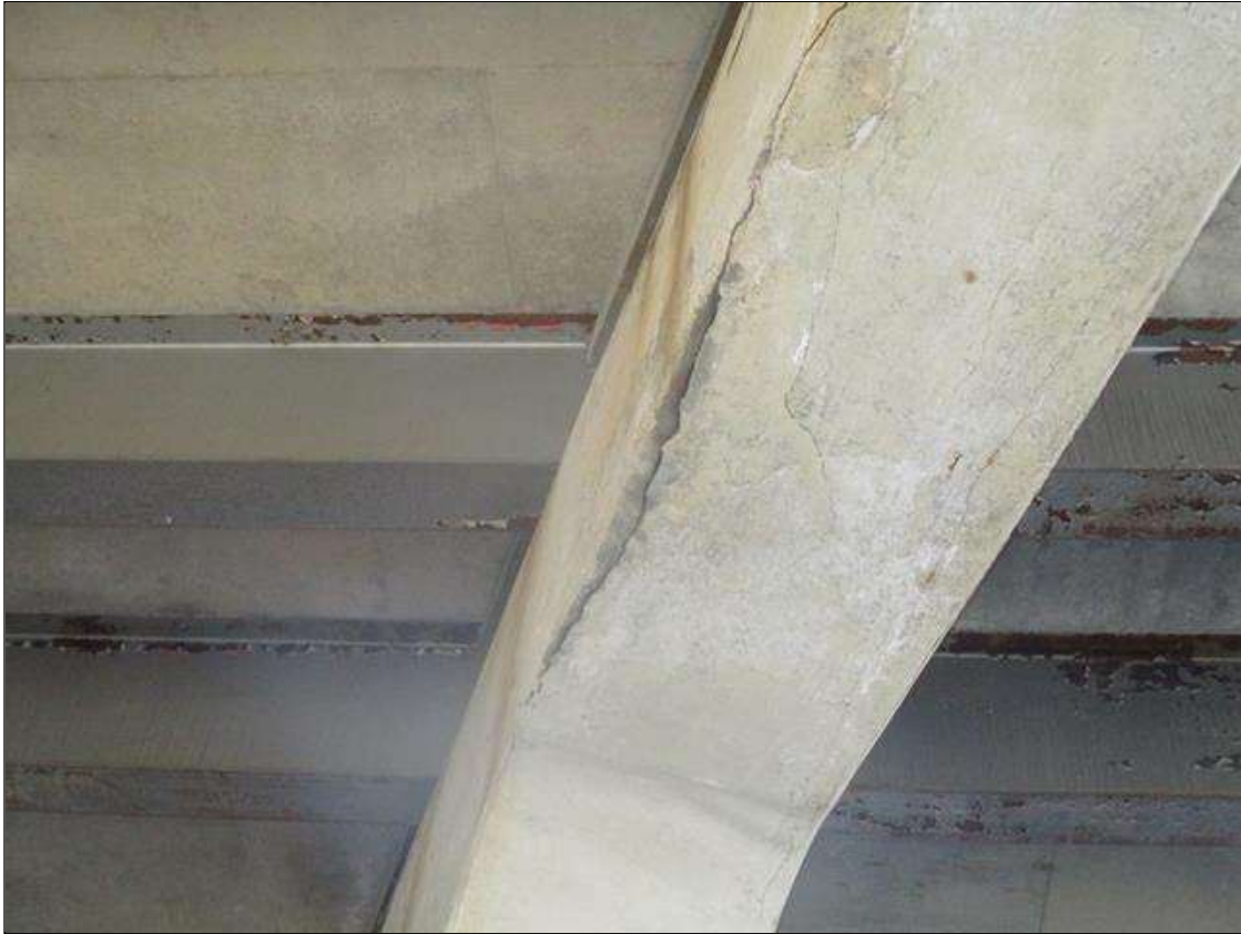
Bent 1 Cap 1: SPALL (2FT L. X 1FT H. X 8IN D.) WITH EXPOSED REINFORCING WITH UP TO 80% SECTION REMAINING IN THE EXPOSED REBAR AT THE BOTTOM EDGE TO THE LEFT OF COLUMN 4, NEAR FACE UNDER BEAM 7 & DELAM (16SF) WITH CRACK UP TO ONE IN WIDE TO TOP & BOTTOM EDGE (DELAM NOT UNDER BEARING) WITH RUST STAINING, NEAR FACE AT BAY 8, FAR FACE SIMILAR & DELAM (16SF) TO TOP & BOTTOM EDGE (DELAM NOT UNDER BEARING) WITH RUST STAINING, FAR FACE AT BAY 6 & DELAM (12SF) TO TOP EDGE (DELAM NOT UNDER BEARING), FAR FACE OVER COLUMN 1
