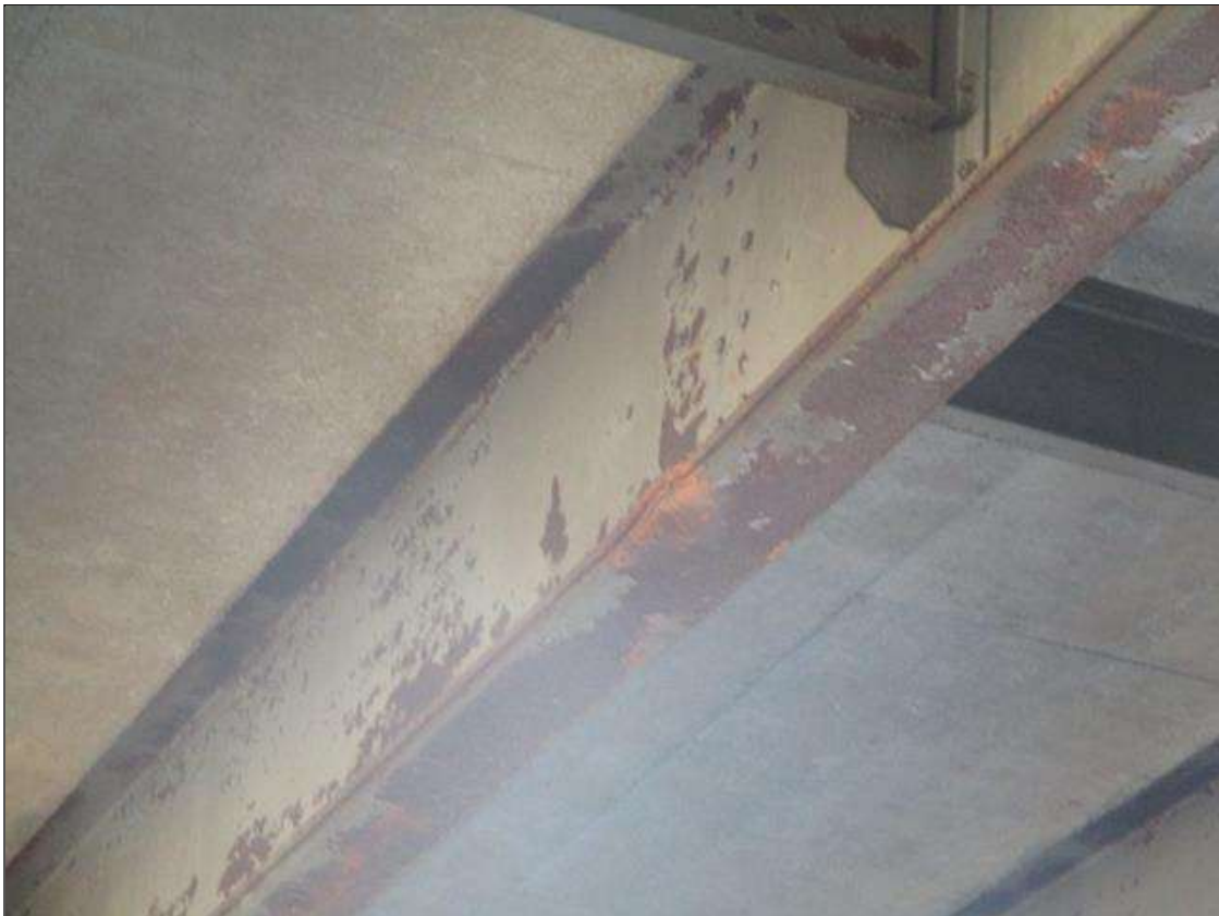
Span 3 Beam 3: IMPACT DAMAGE: 18"L SECTION OF BOTTOM FLANGE AND COVER PLATE BENT UPWARD 1-1/2" AT 24' FROM BENT 3 BEARING. (PAR)
