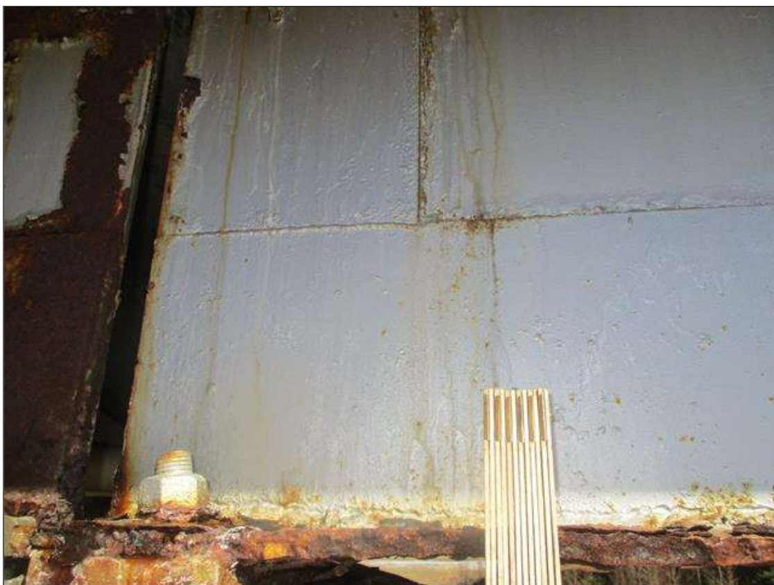
Span 3 Beam 10: BOTTOM FLANGE SECTION LOSS (UP TO 27%, 1/4IN SL, 11/16IN REMAIN) FULL WIDTH FOR 12IN L. AT NEAR END RIGHT SIDE (PAR).
