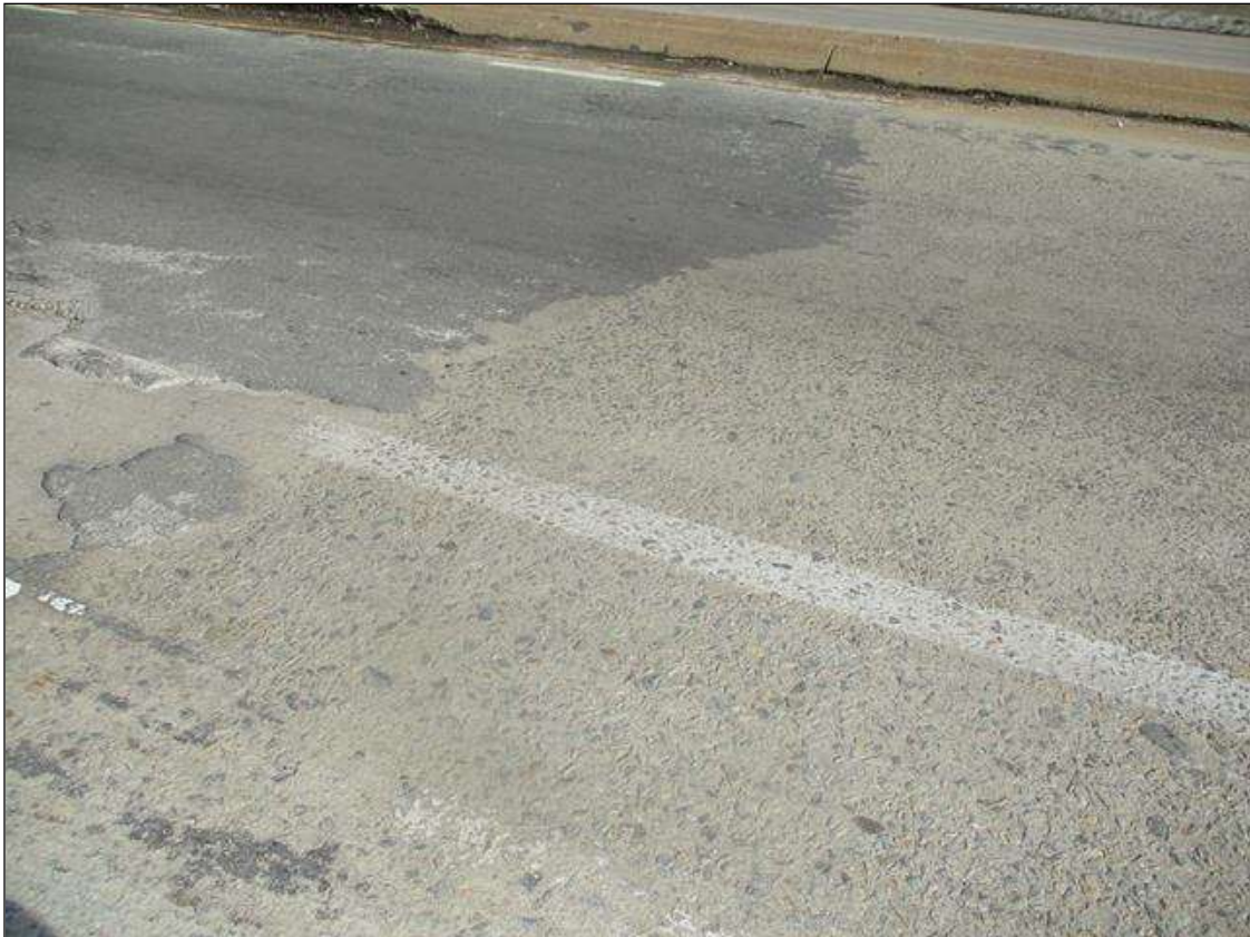
Span 1 Deck: HAIRLINE TO 1/16IN OPEN MAP CRACKING (UP TO FULL WIDTH) THROUGHOUT & WEAR WITH EXPOSED AGGREGATE THROUGHOUT RIGHT LANES
