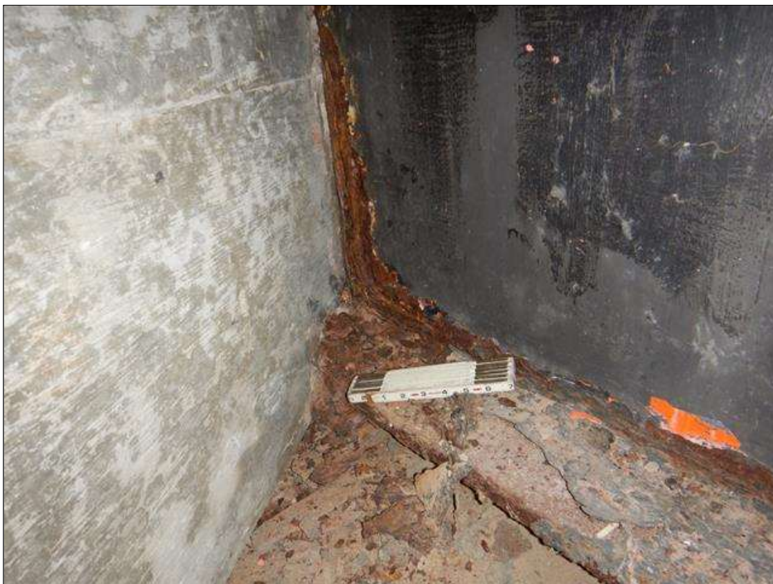
Span 1 Beam 1: at End Bent 1, Rust and Scale no measurable Section Loss in bottom flange and lower web.
