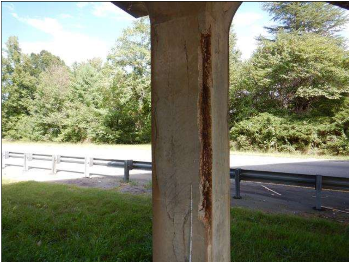
Bent 2 Pile 1: Corner Spall with Exposed Steel Active Corrosion (10' high x 6" x 5",) vertical cracks (1/4" wide x full height) and Delamination in all faces. (PAR)
