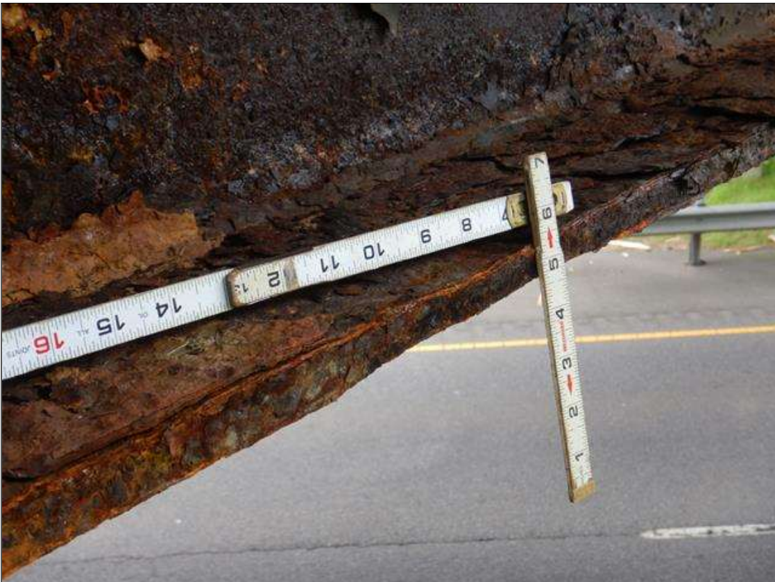
Span 3 Beam 1: BEAM 1, SPAN 3 HAS UP TO 1/8" LOSS ALONG WEB AT PIER 3, 1' HIGH X 1' LONG. ALSO HAS UP TO 1/8" LOSS ALONG BOTTOM FLANGE AT PIER 3, 1' LONG X WIDTH. (PAR)
