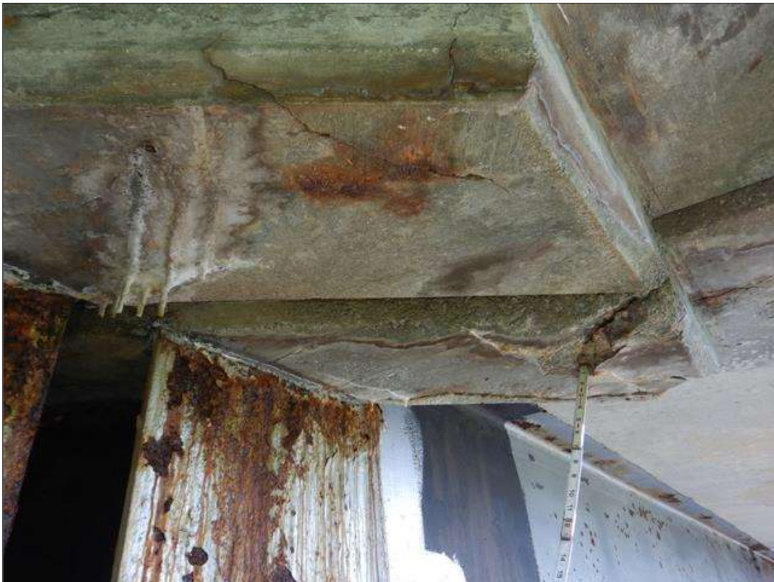
Span 4 Deck: DELAMINATION SPALLED AREA WITH EFFLORESCENCE UNDERSIDE AT BENT 3 OVERHANG 3 FT LONG X 2.5 FT WIDE X 2 IN DEEP
