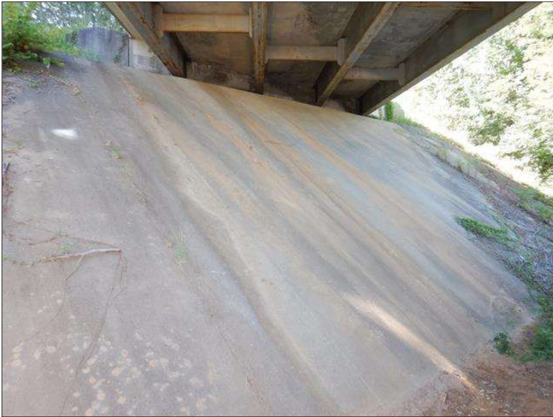
SLOPE PROTECTION, END BENT 1
