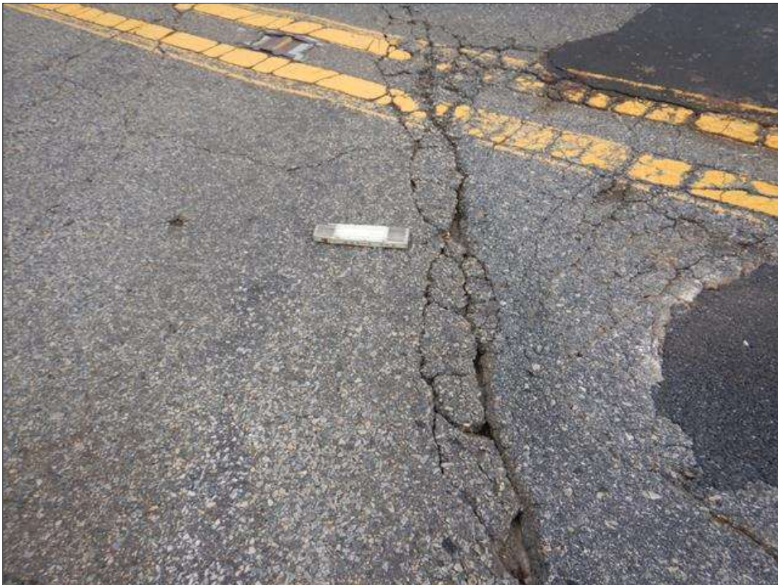
END BENT 1 JOINT HAS TRANSVERSE CRACKING FOR 5 FT WIDE X 1 FT LONG X 2 IN DEEP, AREA OF DETERIORATED ASPHALT
