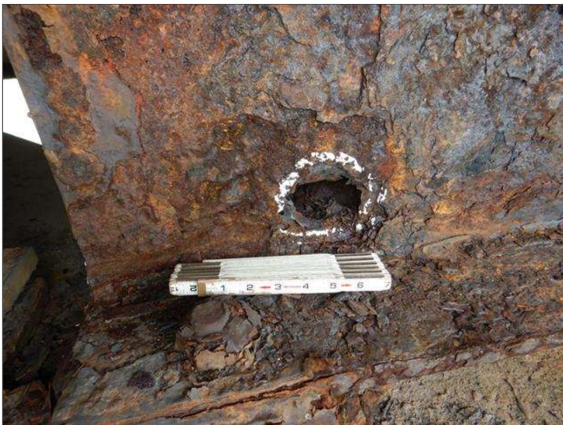
Span 2 Beam 1: DISTORTION FOR 9 IN LONG X 1 IN HIGH AT BOTTOM OF WEB INSIDE OF WEB IS CRACKED. HOLE IN WEB 3 IN IN DIAMETER 9 IN FROM FAR BEARING. (PAR)
