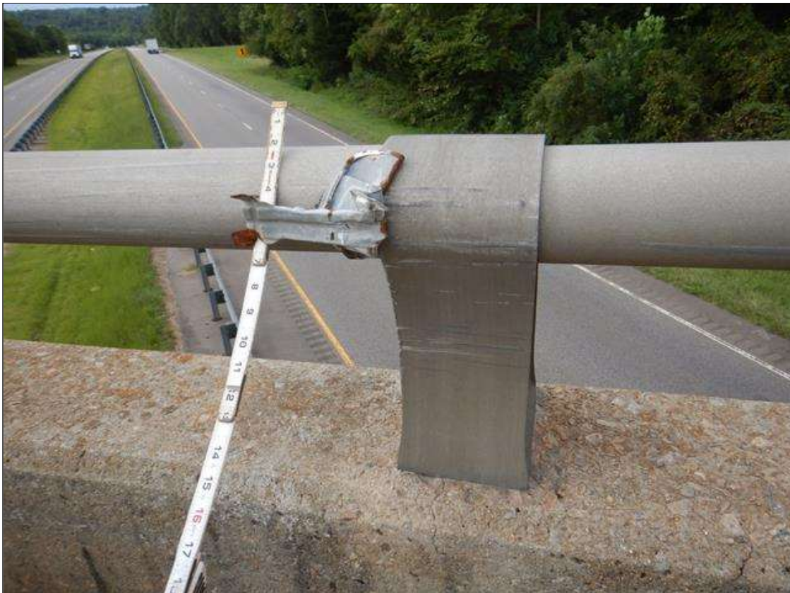
Span 2 Right Bridge Rail: Aluminum Post #9, scrapes to traffic side. Connections intact, post functioning as intended.
