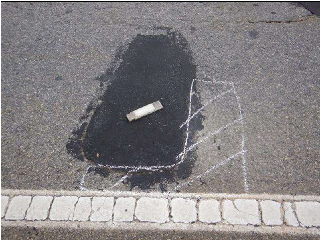
Span 2 Wearing Surface: DELAMINATED AREA IN MIDDLE OF SPAN 2 IN RIGHT TRAVEL LANE 2 FT X 2 FT. TYPICAL FOR MOST PATCHED POTHOLES
