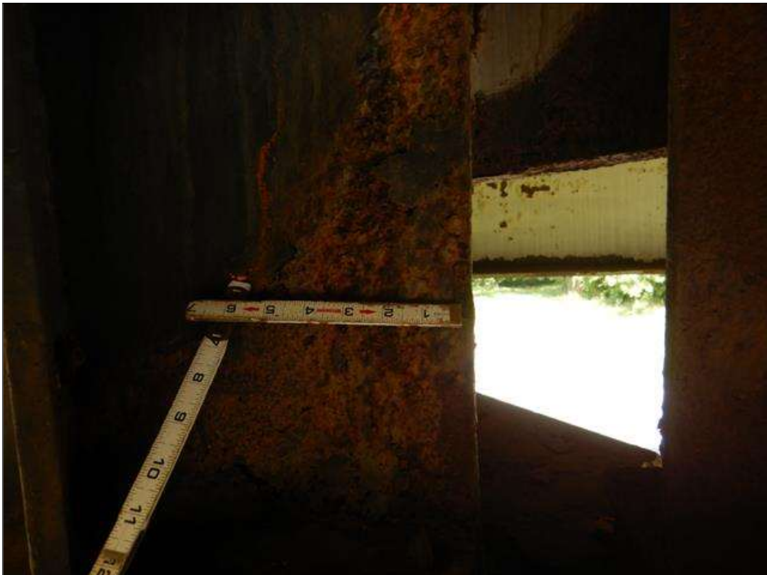
Span 2 Beam 3: at Bent 2, Active Corrosion & Section Loss in Bottom flange (7/16" Remaining full width to 5" wide x 2' long,) lower web, (5/16" Remaining full height x 10" long then 3" high x 6" long.) (PAR)
