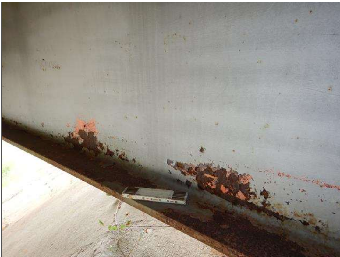
Span 1 Beam 4: Surface Corrosion/ Freckled Rust in flanges and web along length of beam.
