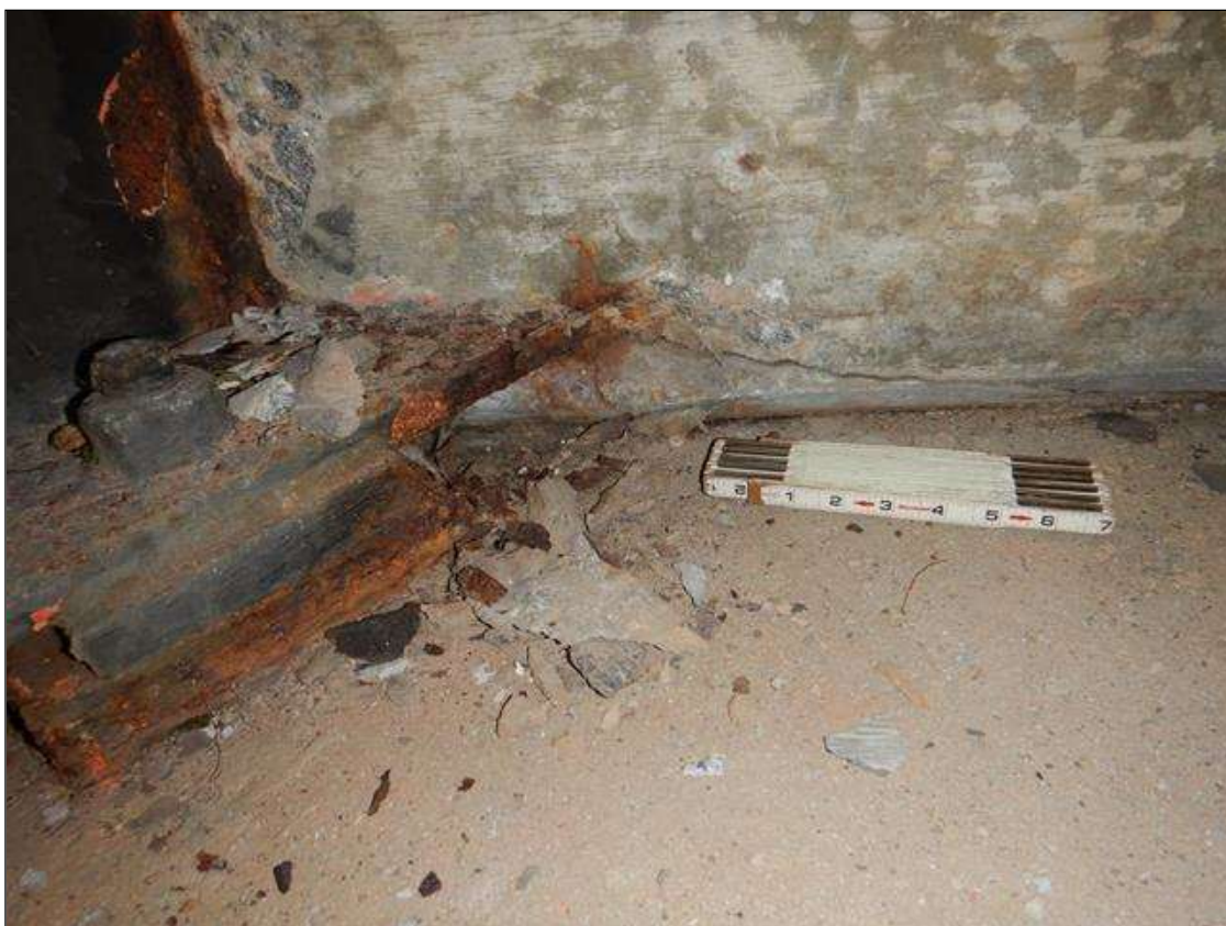
Span 1 Beam 3: AREA WHERE BEAM 3 GOES INTO END BENT 1 CRACKING UP TO 1 FT LONG AND SMALL SPALL UP TO 3 IN DIAMETER X 3/4 IN DEEP
