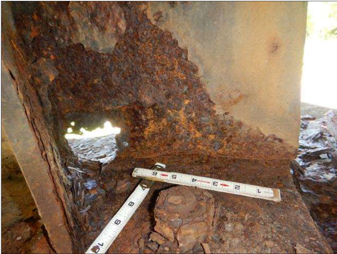
Span 3 Beam 1: 6" LONG X 1/4" WIDE CRACK IN BOTTOM FLANGE EXTENDS INTO WEB VERTICALLY IN BEAM 1 SPAN 3 LOCATED ON SOUTH SIDE OF BEAM. (PAR)
