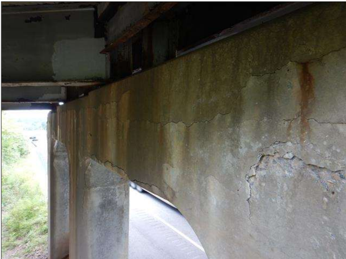
Bent 3 Cap 1: DELAMINATION AND CRACKING ALONG FULL WIDTH OF EAST FACE BENT 3
