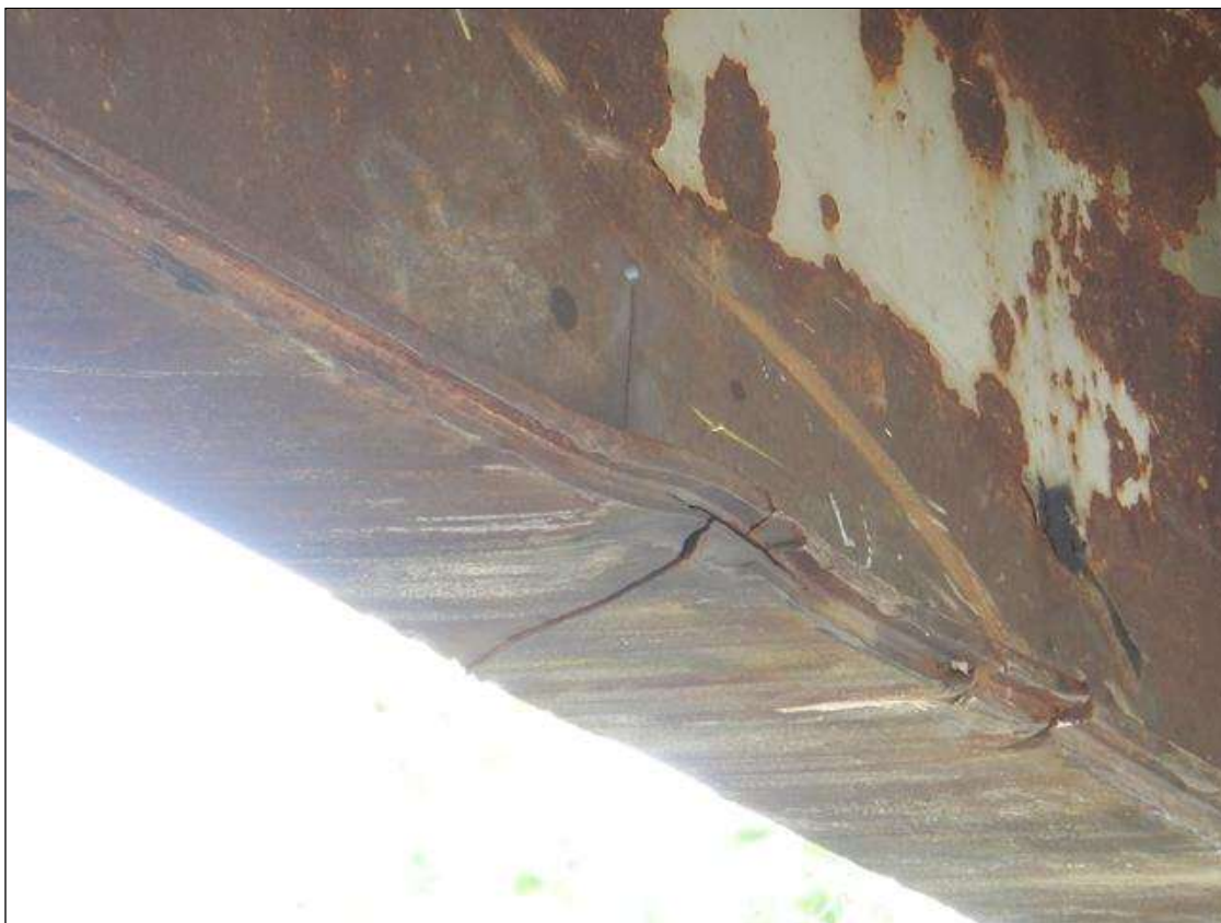
Span 3 Beam 1: 6" LONG X 1/4" WIDE CRACK IN BOTTOM FLANGE EXTENDS INTO WEB VERTICALLY IN BEAM 1 SPAN 3 LOCATED ON SOUTH SIDE OF BEAM. (PAR)
