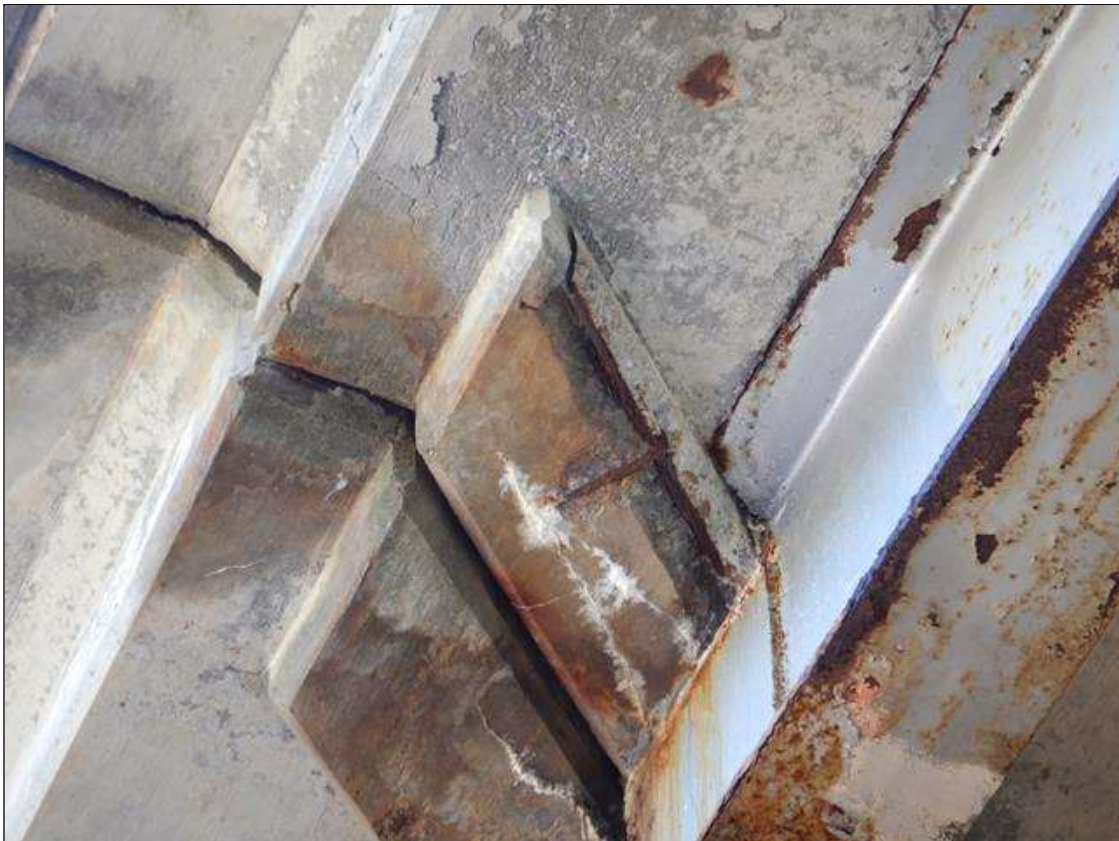
Span 1 Beam 1: RC end diaphragm at Bent 1, left overhang, Spall with Exposed Steel (28" x 6" x 3" deep.)
