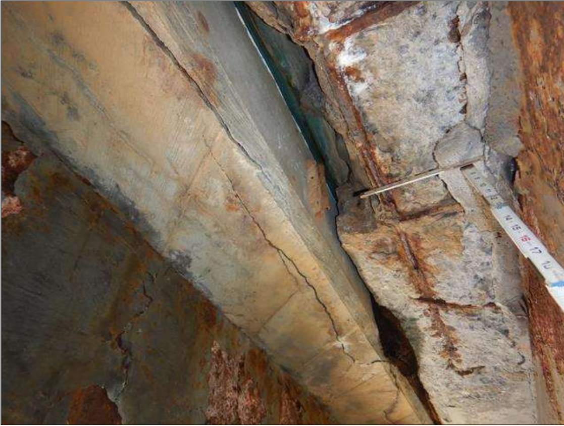
Span 1 Deck: SPALL IN DECK UNDERSIDE IN BAY 3 FOR 6 FT LONG X 1 FT WIDE X UP TO 6 IN HIGH. 80% SECTION REMAINING IN EXPOSED REBAR
