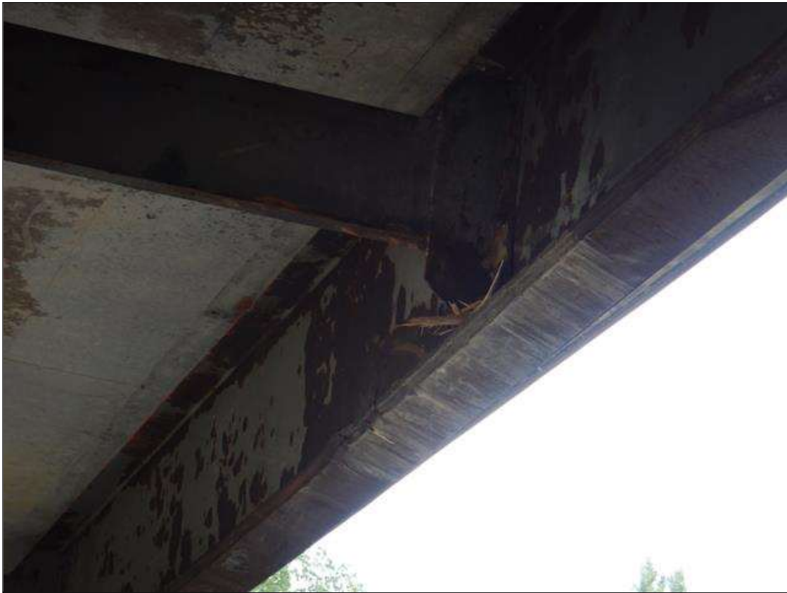
Span 3 Beam 1: Impact damage due to high load, with Out of plane bending in bottom flange and web. Point of impact located approximately 18' from Bent 3, above US220 North.
