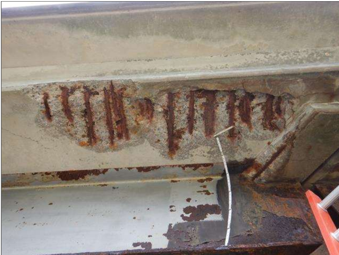
Span 3 Deck: Underside of deck at Bent 2, left overhang, Spall with Exposed Steel/ Delamination, (6' x 2' x 2" deep,) with loose concrete above mowable grass shoulder. (PAR)
