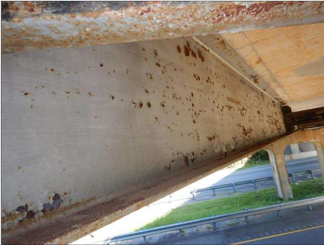
Span 1 Beam 2: 53 Feet of Corrosion: Section loss is evident or pack rust is present but does not warrant structural review. RIGHT SIDE SHOWN
