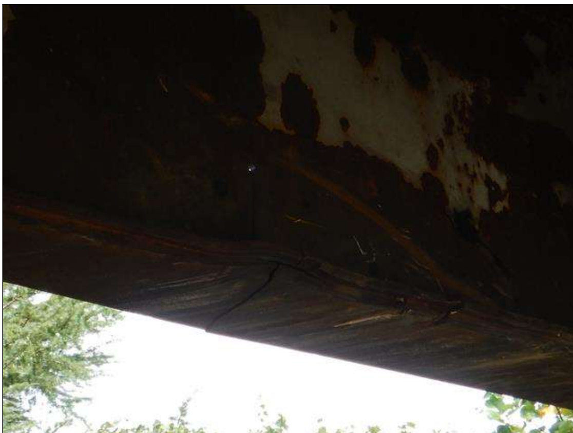
Span 3 Beam 1: 6" LONG X 1/4" WIDE CRACK IN BOTTOM FLANGE EXTENDS INTO WEB VERTICALLY IN BEAM 1 SPAN 3 LOCATED ON SOUTH SIDE OF BEAM. (PAR)
