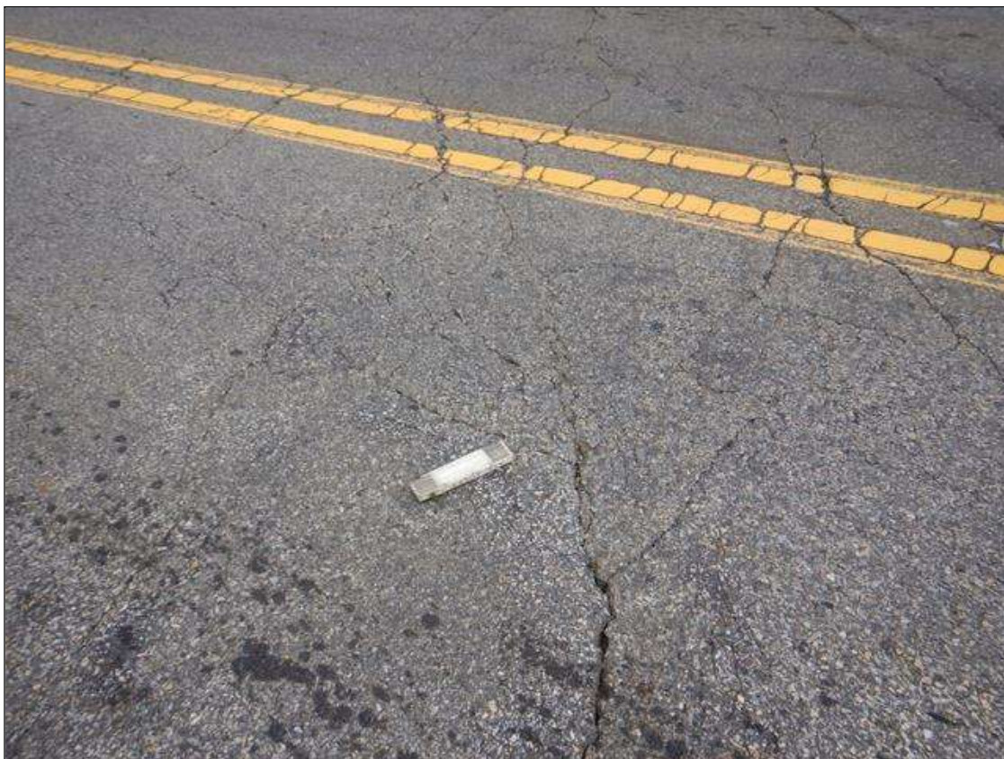
WEST APPROACH HAS HEAVY AREA OF MAP CRACKING UP TO 1/2 IN WIDE
