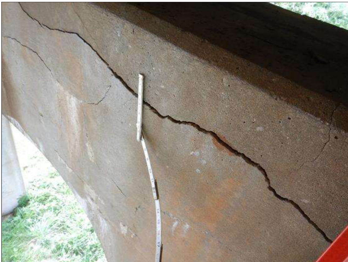
Bent 2 Cap 1: HORIZONTAL CRACKING UP TO 1/4" AND DELAMINATION ALONG LENGTH OF BOTH FACES
