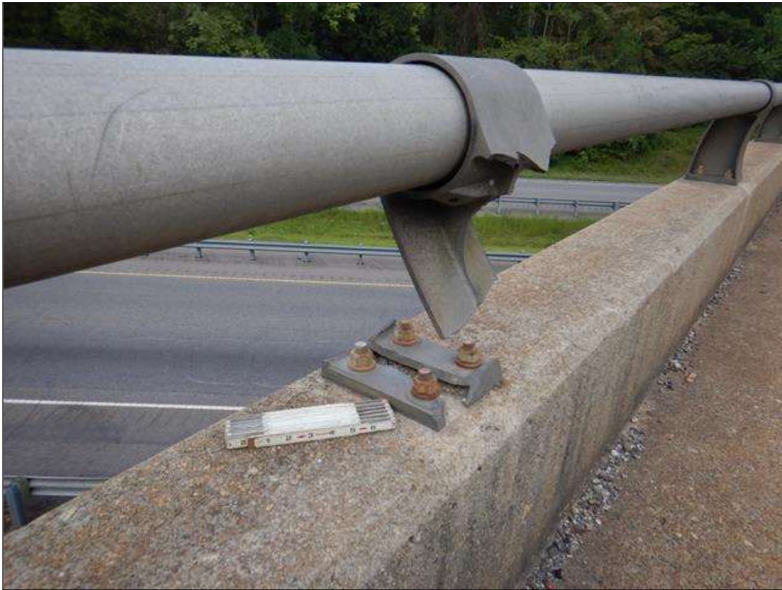
Span 4 Right Bridge Rail: ALUMINUM POST # 4 IS BROKEN AND COMPLETELY DETACHED FROM ITS BASE. (PAR)
