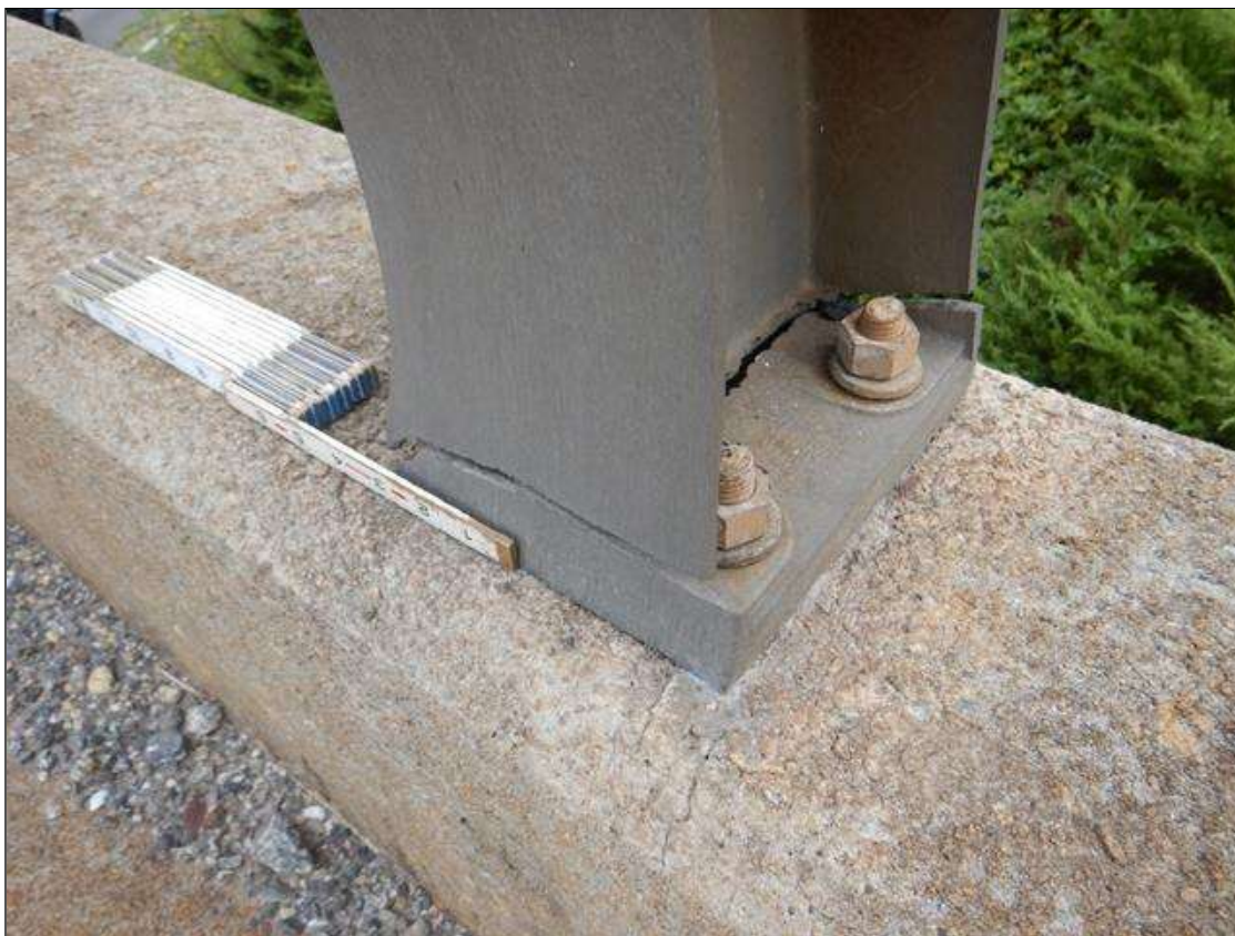
Span 4 Left Bridge Rail: ALUMINUM POST # 5 IS CRACKED AT BASE. (PAR)
