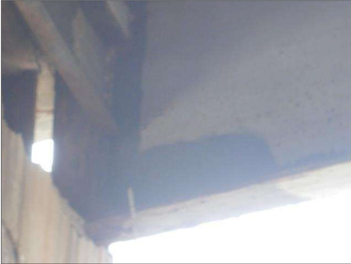
Span 2 Beam 4: at Bent 2, Active Corrosion & Section Loss in Bottom flange in front of bearing (5/8" Remaining full width x 12" long,) lower web, (5/16" Remaining 12" high x 10" long,) Upper Web (5/16" Remaining 12" high x 10" long,) Web stiffener / diaph connection plate (5/8" Remaining 5" x 4".) (PREVIOUS PAR VISUALLY INSPECTED DUE TO UNSAFE ROAD CONDITIONS FOR LADDER SETUP)
