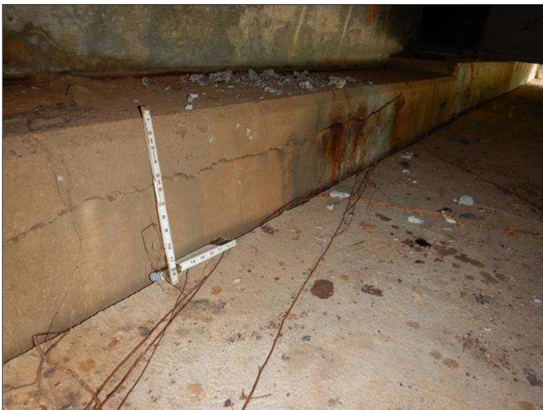
End Bent 1 Cap 1: CRACKING GOING ACROSS CAP SEAT FOR FULL WIDTH UP TO 1/2 IN WIDE WITH AREAS OF DELAMINATION
