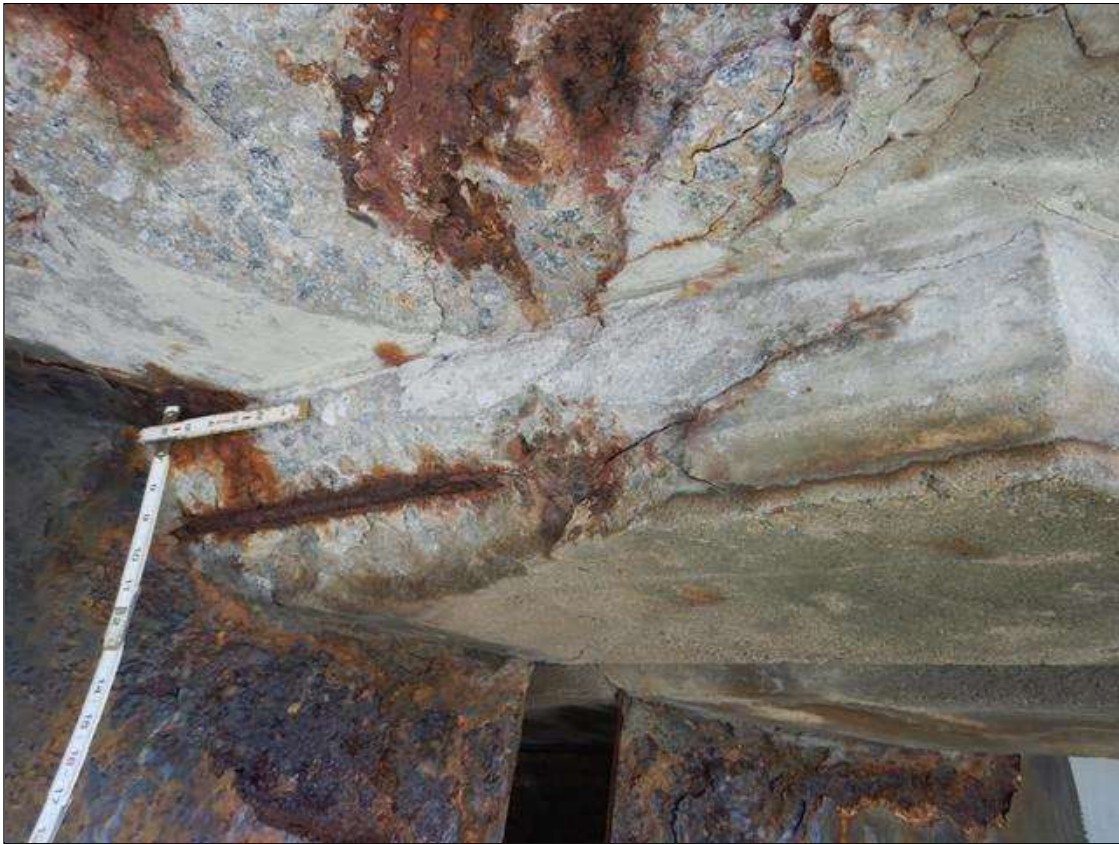
Span 3 Deck: RC DIAPHRAGM ON LEFT OVERHANG UNDERSIDE DECK HAS SPALL WITH EXPOSED REBAR FOR 2 FT WIDE X 6 IN HIGH X 5 IN LONG. 80% SECTION REMAINING ON EXPOSED REBAR.
