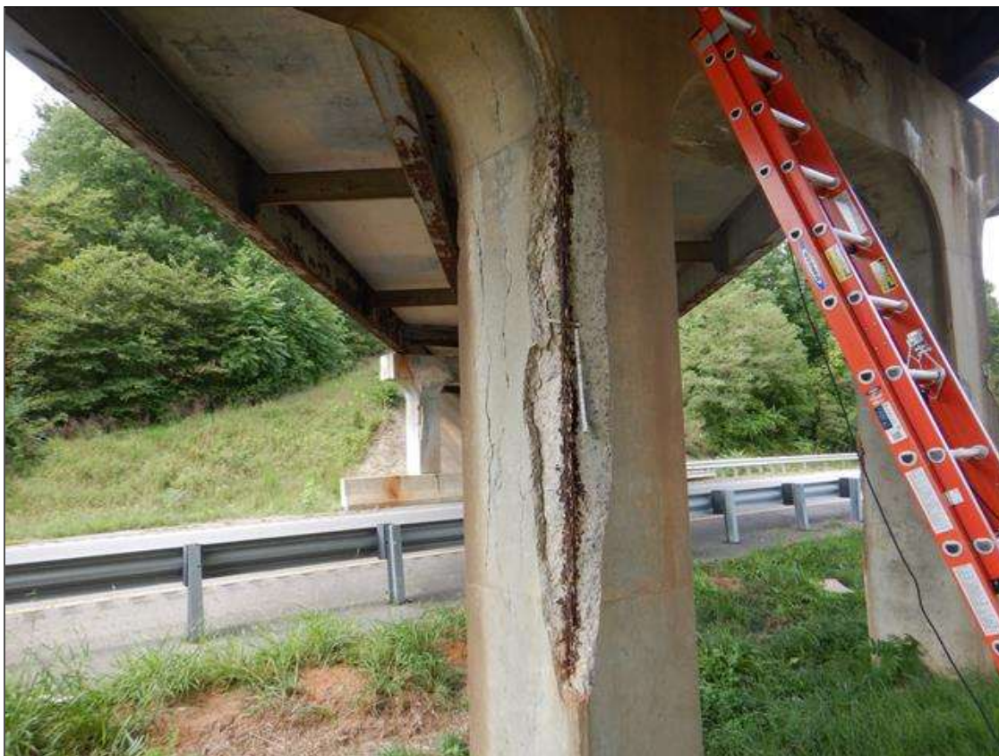
Bent 2 Pile 2: Corner Spalls with Exposed Steel (Active Corrosion no measurable Section Loss,) (up to 8' high x 1 FT LONG x 1 FT,) vertical cracks (1/4" wide x full height) and Delamination in all faces. 80% SECTION REMAINING ON EXPOSED REBAR. (PAR)
