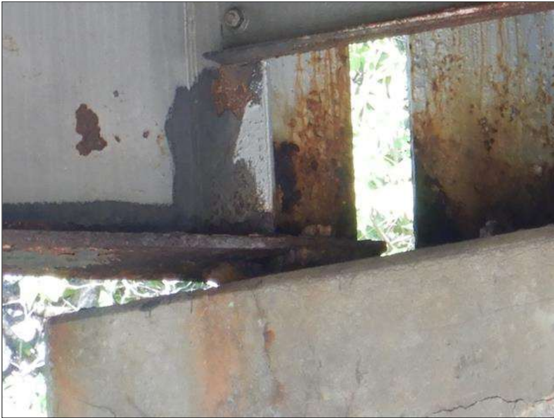
Span 2 Beam 4: at Bent 1 LEFT FACE, beginning 1' from beam end, Active Corrosion & Section Loss in lower web (1/4" Remaining 3" high x 22' long,) right bottom flange (13/16" Remaining 5" wide x 22' long.) (PAR VISUALLY INSPECTED)
