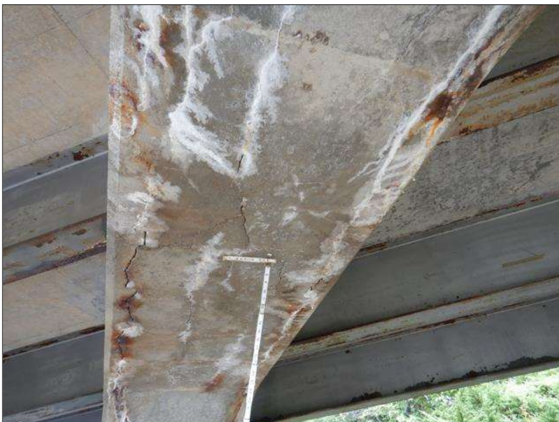
Bent 3 Cap 1: CRACKS FULL WIDTH UNDERSIDE CAP BETWEEN PILES 2 AND 3 WITH HEAVY EFFLORESCENCE BUILDUP
