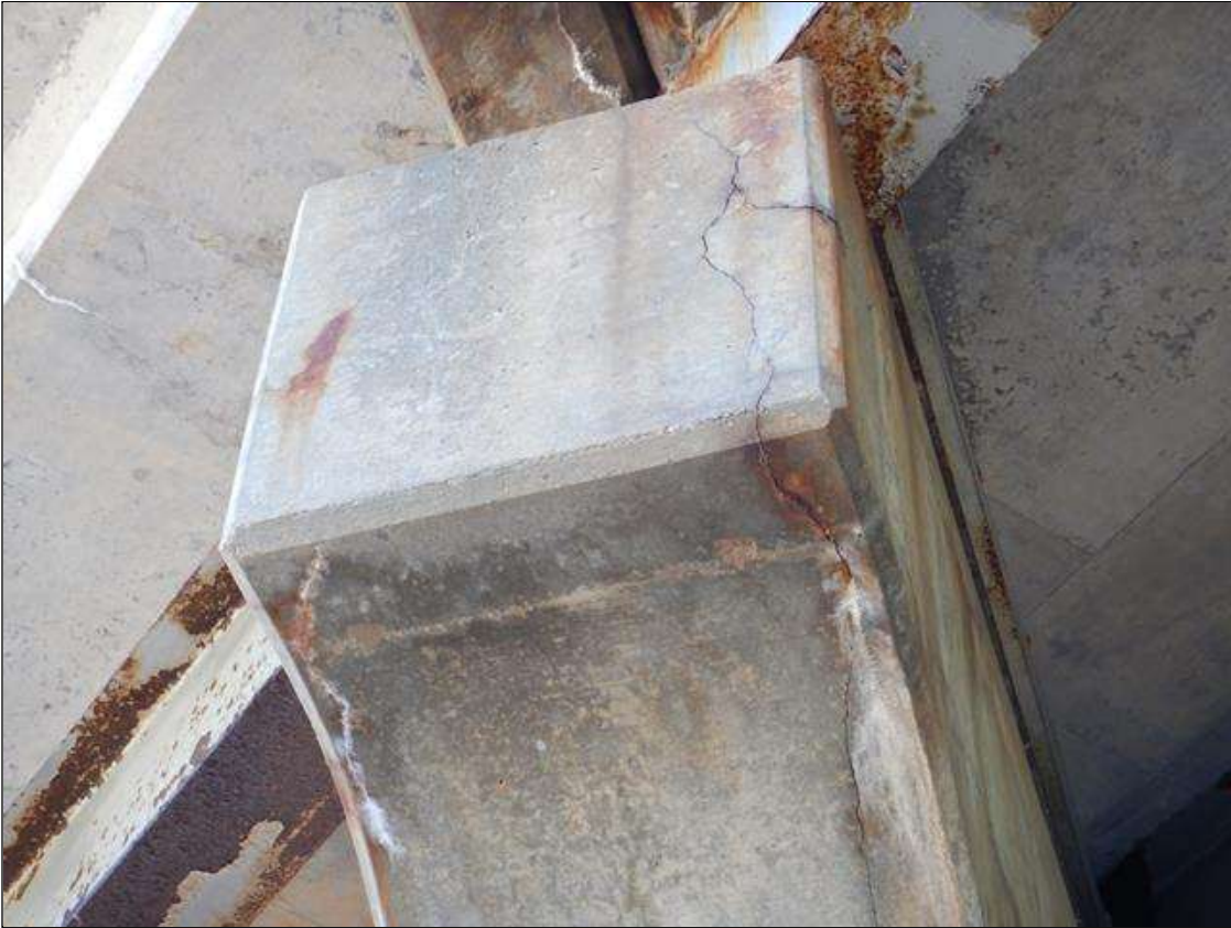
Bent 1 Cap 1: North end of cap, West and East faces, Map cracks (1/16" wide) with rust stains and efflorescence, Delamination 7' long x up to 32" high x 3" wide at top.)
