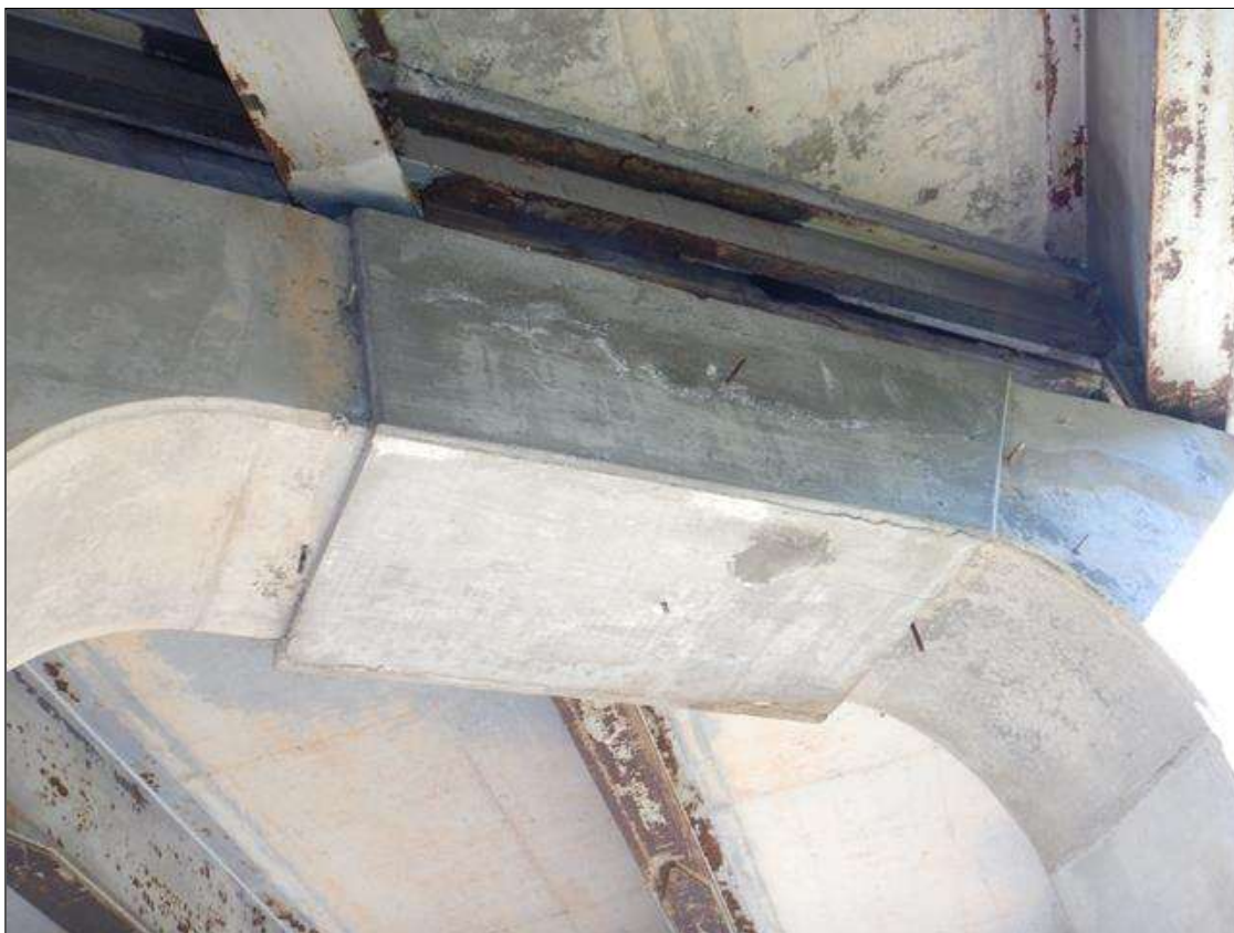
Bent 1 Cap 1: (Previous Repair:) Top of Cap, From South end to bay 3, beneath Bearings for Beam 4, Spans 1 & 2, Sound concrete repair with vertical shrinkage crack (1/64" wide) on west face. Bay 3, Sound concrete repair to full circumference, west face near top has horizontal shrinkage crack (1/64" wide x 5' long.)
