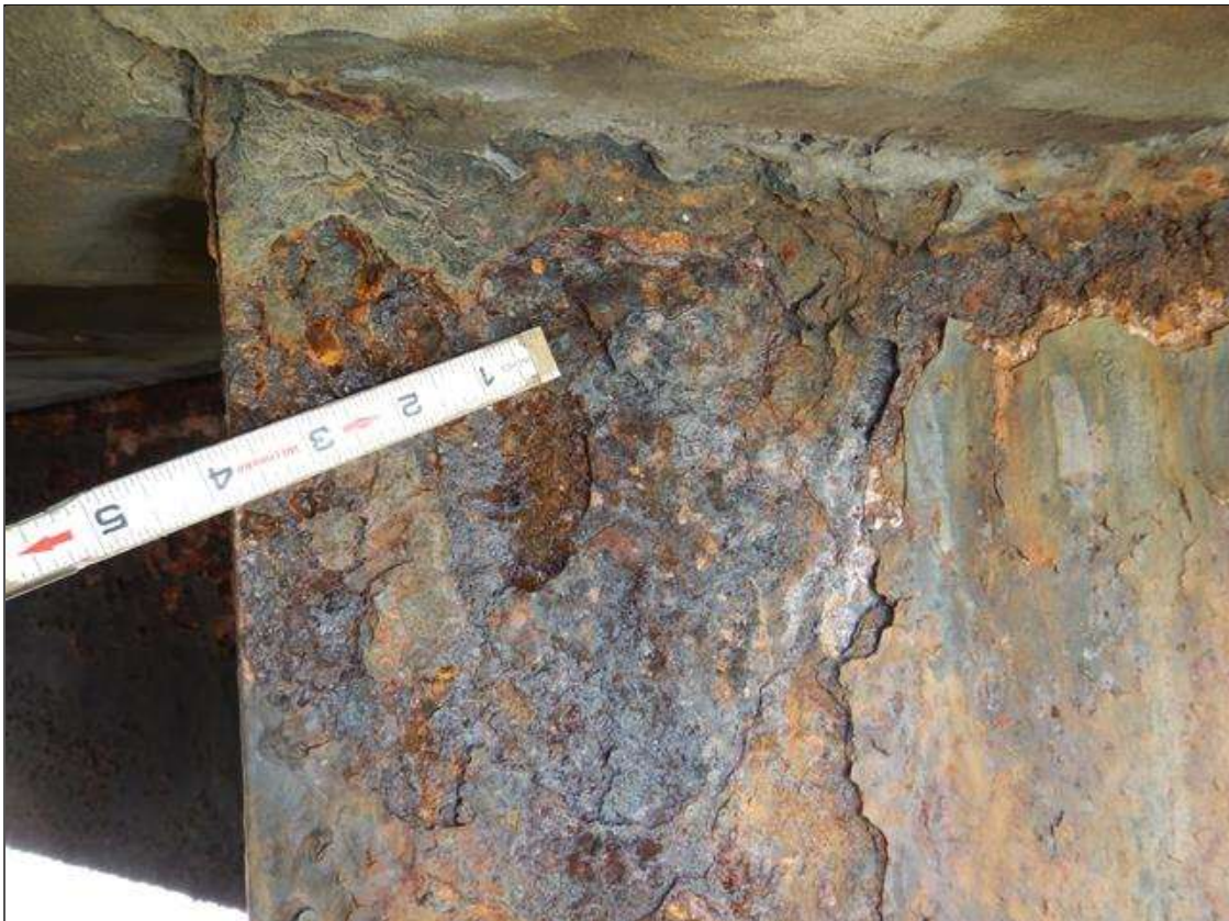
Span 2 Beam 1: at Bent 2, Active Corrosion & Section Loss in Lower web (1/16" Remaining 6" high x 2' long) Upper web (1/8" Remaining 18" long x 8" high,) Bottom Flange (5/8" to 3/4" Remaining full width x 18" long.) (PAR)
