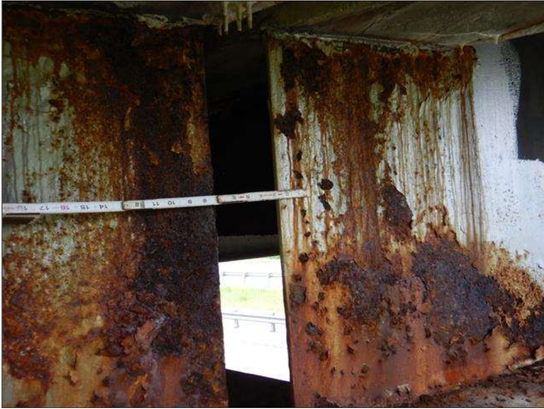
Span 4 Beam 1: HEAVY CORROSION AT BEAM ENDS 1 AND 2 AT BENT 3
