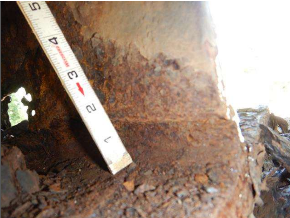
Span 3 Beam 1: 6" LONG X 1/4" WIDE CRACK IN BOTTOM FLANGE EXTENDS INTO WEB VERTICALLY IN BEAM 1 SPAN 3 LOCATED ON SOUTH SIDE OF BEAM. (PAR)
