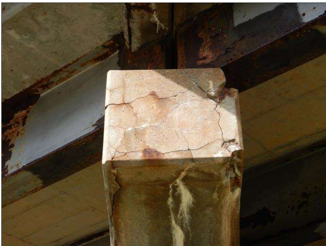
Bent 2 Cap 1: SOUTH SIDE OF CAP END HAS DELAMINATION WITH SPALL FOR 6 IN DIAMETER 1.5 IN DEEP WITH 90% SECTION REMAINING ON EXPOSED REBAR.
