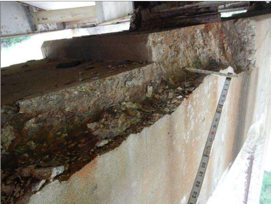
Bent 2 Cap 1: Top corners of cap, east and west faces, in bay 3 to south end, Spall with Exposed Steel (Active Corrosion no measurable Section Loss) and Delamination 6' long x up to 12" high x up to 10" wide.). (PAR)
