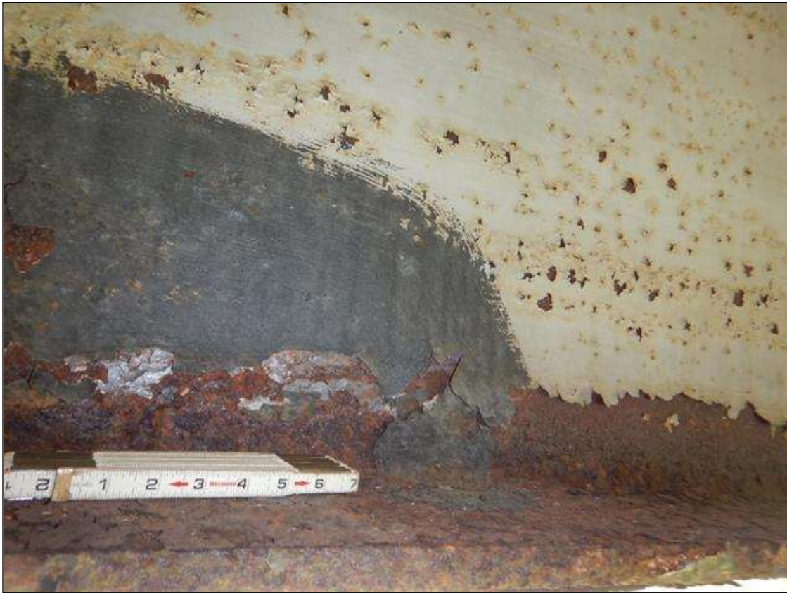
Span 2 Beam 4: at Bent 2, beginning 12" from beam end, Active Corrosion & Section Loss in lower web, (1/2" Remaining 3" high x 4' long,) Bottom Flange (3/4" Remaining 5" wide x 4' long.) (PAR)
