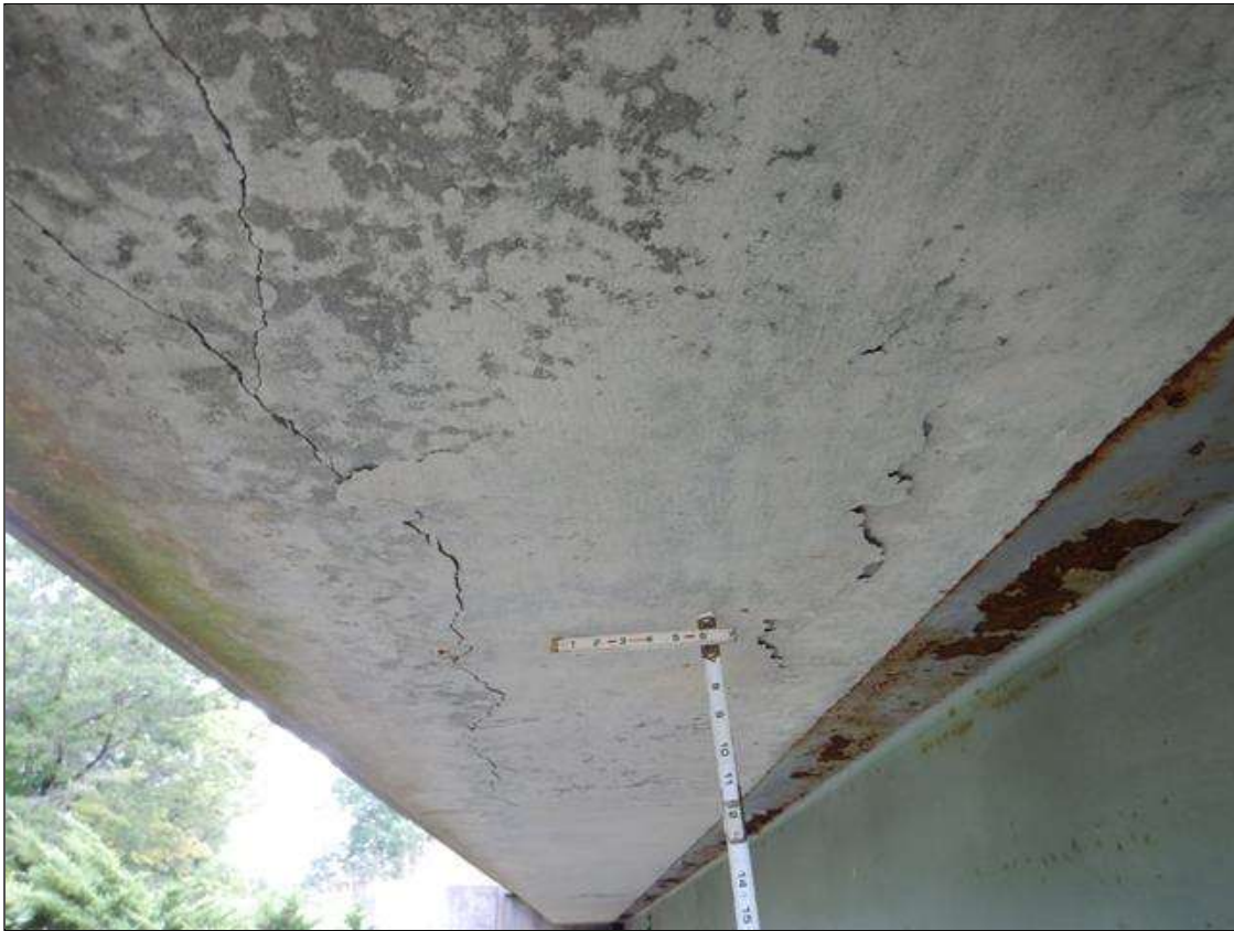
Span 4 Deck: DELAMINATED AREA IN DECK UNDERSIDE GOING FROM BENT 3 TOWARD END BENT 2 FOR 10 FT LONG X 2.5 FT WIDE
