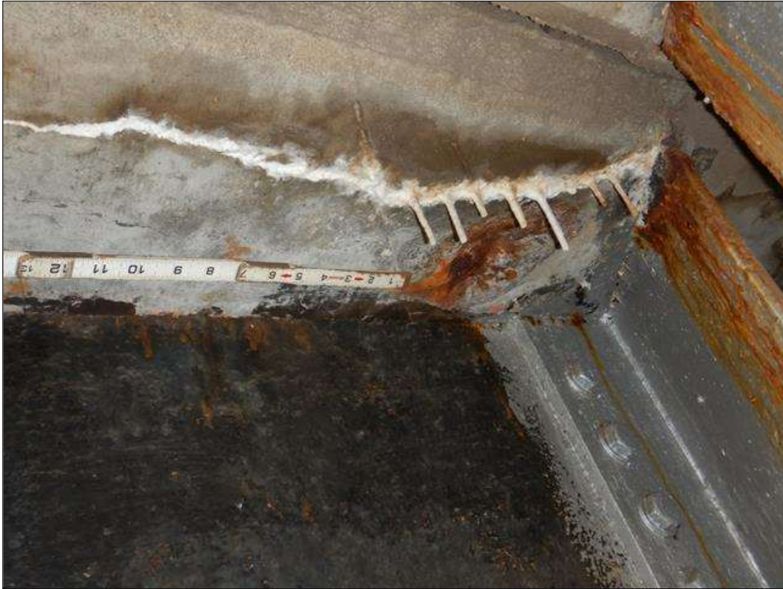
Span 3 Deck: UNDERSIDE DECK AT BENT 3 IN BAY 3 HAS CRACKING UP TO 1/32 IN WITH EFFLORESCENCE. 6 IN DIAMETER SPALL X 1 IN DEEP WITH EXPOSED REBAR. 90% SECTION REMAINING IN EXPOSED REBAR
