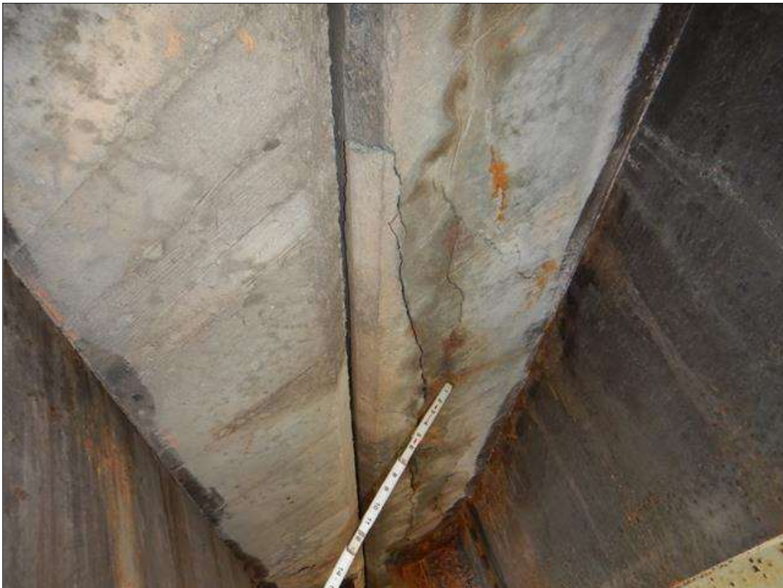
Span 2 Deck: UNDERSIDE DECK HAS CRACKING UP 1/4 IN WIDE X 5 FT LONG IN BAY 1, SIMILAR IN OTHER BAYS
