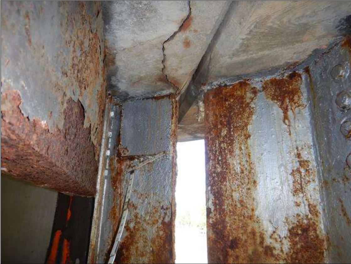
Span 1 Beam 1: (Previous repair:) at Bent 1, right side of Web, Steel plate (1/2" t. x 9" x 9") welded at top on end of beam. Left side, steel plate welded (1/2" x full height x 2' long). Surface Corrosion/Freckled Rust in web below.
