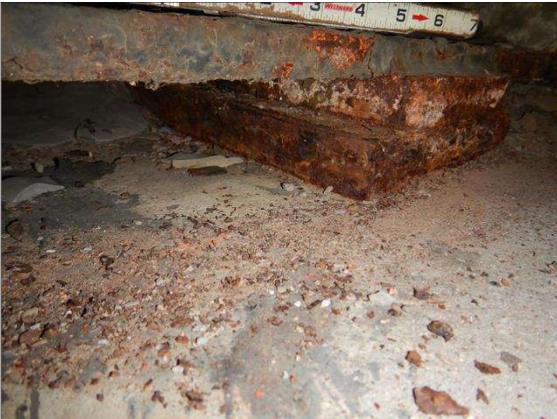
Span 4 Near Bearing: Active Corrosion & Section Loss (1-1/4" Remaining) in plates. ALL OTHER BEARING PLATES AT END BENT 2 ARE SIMILAR
