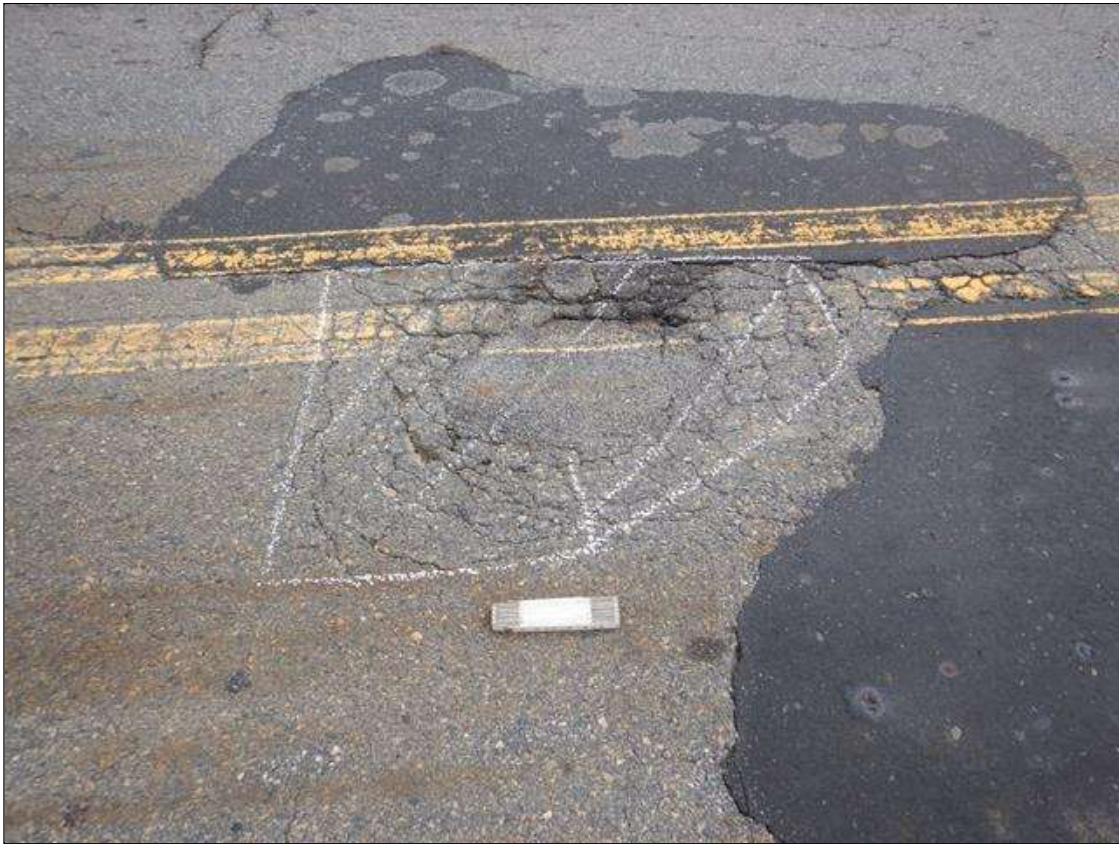
Span 3 Wearing Surface: DELAMINATED SPALLED AREA IN MIDDLE OF SPAN 3 CENTER LINE FOR 4 FT LONG X 3 FT WIDE X UP TO 1 IN DEEP. POTHOLES HAVE TYPICAL PERIMETER AREA OF DELAMINATION
