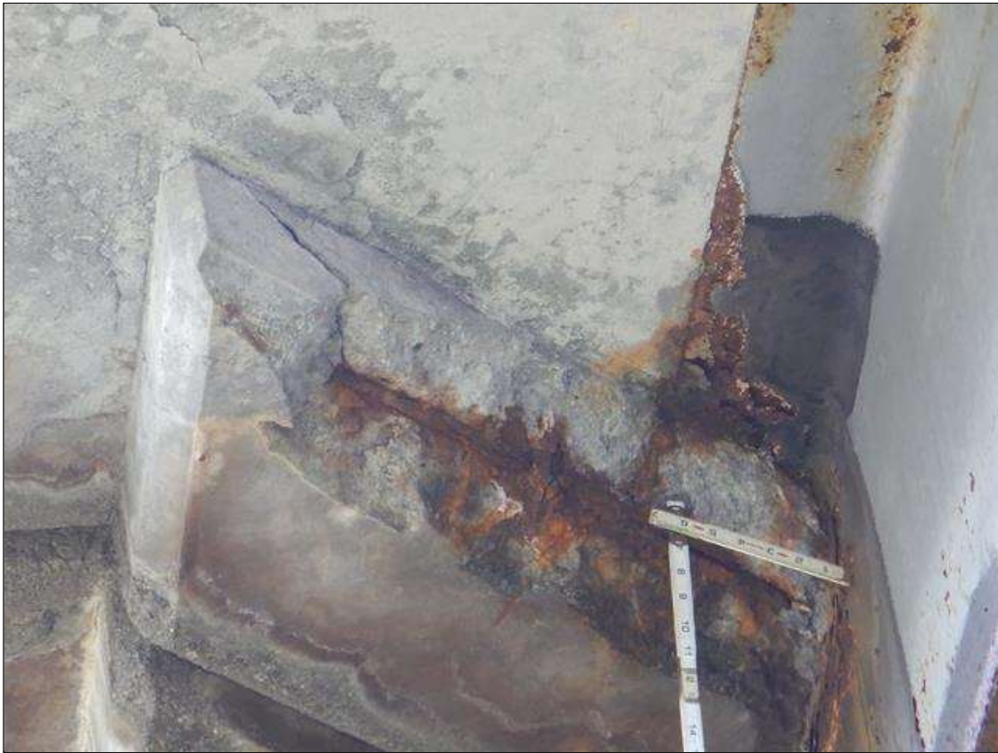
Span 2 Beam 1: RC DIAPHRAGM AT BENT 3 IN SPAN 2 HAS SPALLED AREA 2 FT WIDE X 1 FT LONG X 6 IN HIGH WITH EXPOSED REBAR. 80% SECTION REMAINING IN EXPOSED REBAR
