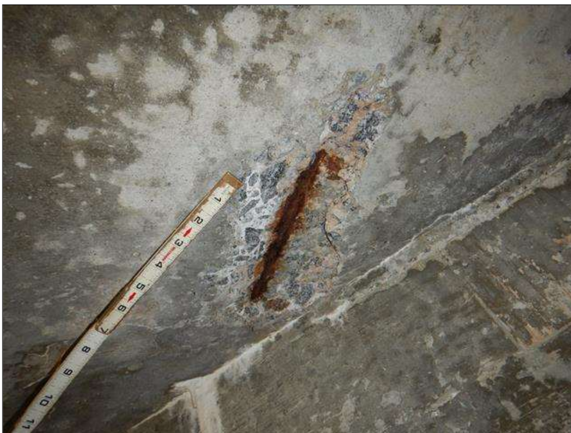
End Bent 1 Abutment: DELAMINATION AND SPALLED AREA IN BAY 3 1 FT DIAMETER X 1 IN DEEP WITH EXPOSED REBAR, 90% SECTION REMAINING IN EXPOSED REBAR
