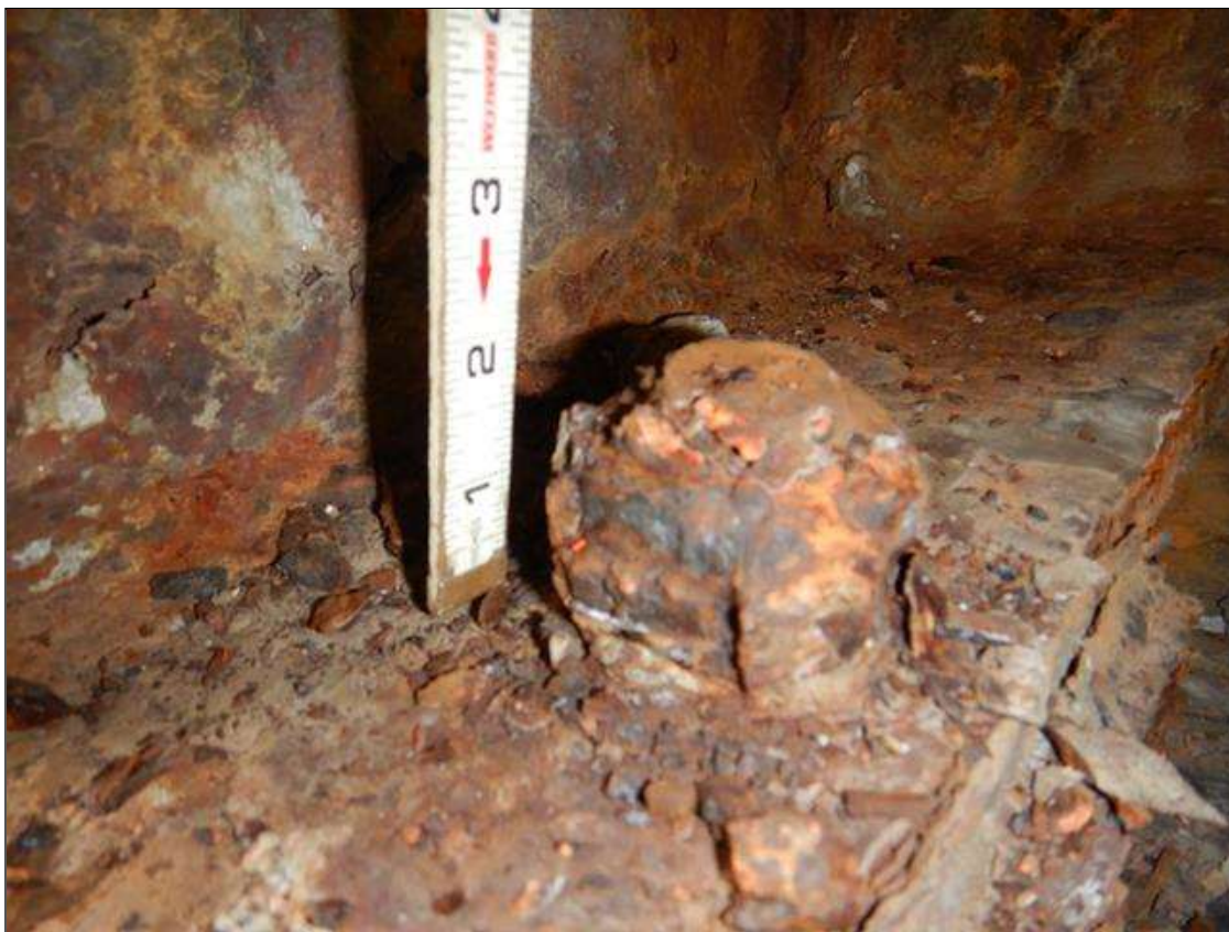
Span 3 Far Bearing: LEFT SIDE ANCHOR BOLT NUT IS CORRODED WITH 80% SECTION REMAINING
