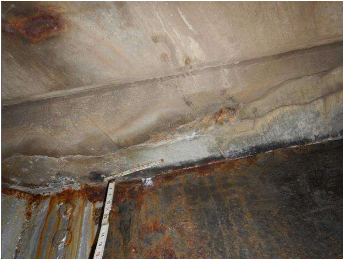
Span 3 Deck: DELAMINATED AREA WITH SPALLING IN DECK UNDERSIDE AT BENT 3 IN BAY 1 WITH CRACKS UP TO 1/8 IN WIDE
