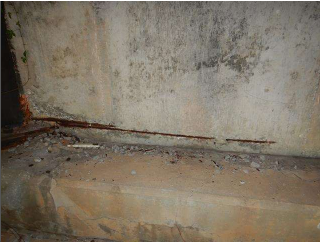
End Bent 2 Abutment: DELAMINATED SPALLED WITH EXPOSED REBAR AREA IN BAY 2 NEXT TO BEAM 2 5 FT WIDE X 6 IN HIGH X 1.5 IN DEEP. 80% SECTION REMAINING IN EXPOSED REBAR. (PAR)
