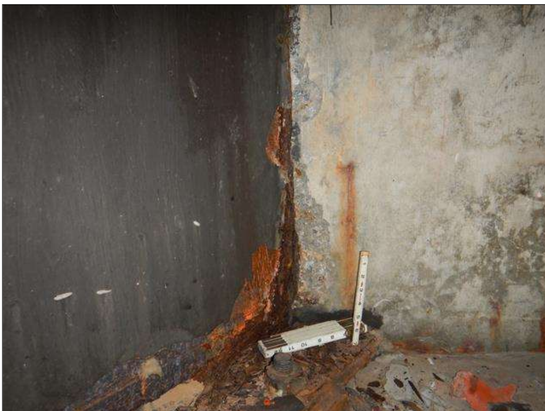
End Bent 2 Abutment: SPALLED AREA IN BAY 1 1.5 FT HIGH X 3 IN WIDE X 1 IN DEEP ALONG RIGHT SIDE OF BEAM 1, NO EXPOSED REBAR
