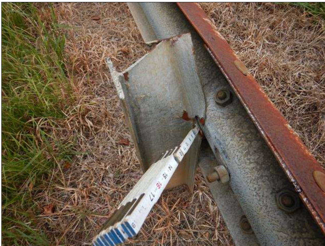
THIRD POST FROM END BENT 1 ON RIGHT GUARDRAIL IS DAMAGED AND DETACHED FROM RAIL. (PAR)
