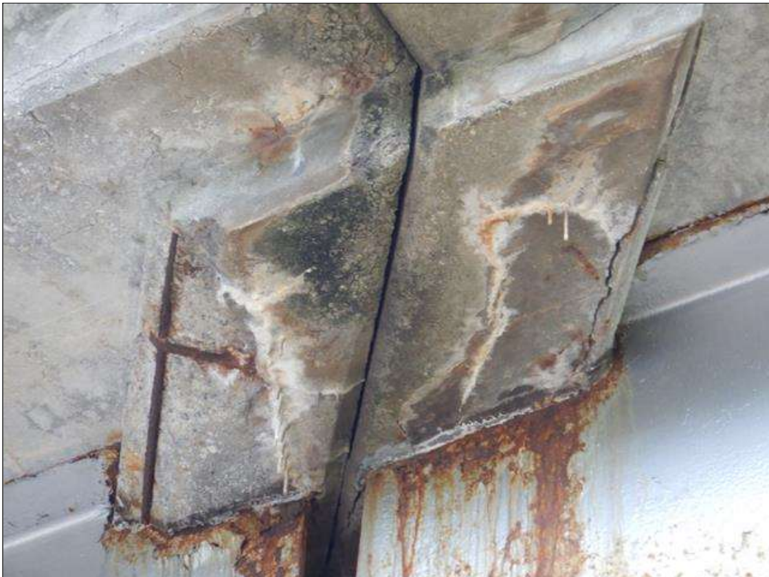
Span 4 Beam 4: RC end diaphragm at Bent 3 IN SPAN 4 right overhang, cracks (1/2" wide) with efflorescence buildup and rust stains.
