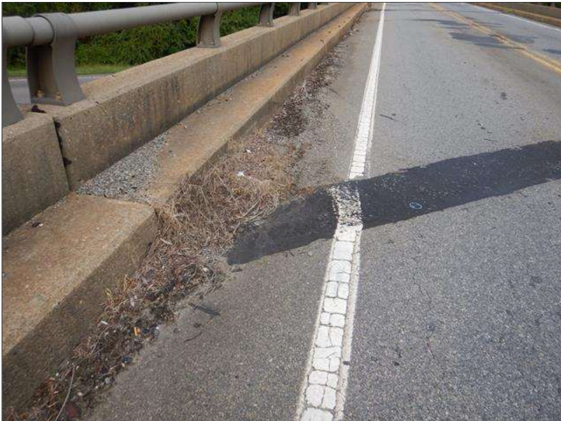
RIGHT BRIDGE RAIL HAS MODERATE DEBRIS IMPACTION THROUGHT ALL SPANS, SPAN 3
