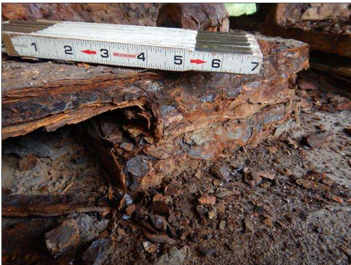
Span 4 Near Bearing: 1 Each of Corrosion: Freckled rust. Corrosion of the steel has initiated.
