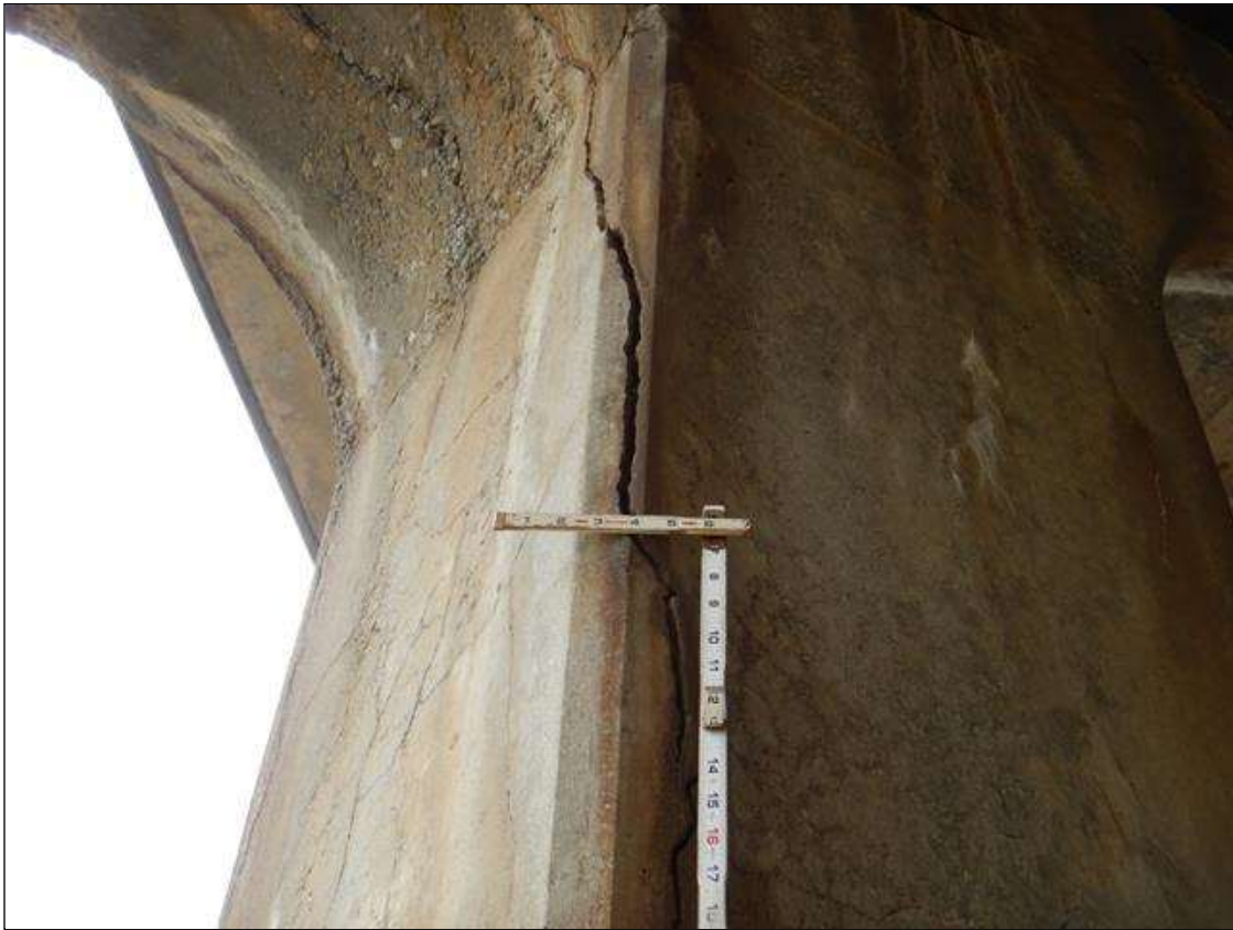
Bent 3 Pile 3: Vertical cracks (1/4" wide) with efflorescence and Delamination (imminent spalling) West face, full height x full width, and east face at 10' below cap (2' wide x 3' high.) (PAR)
