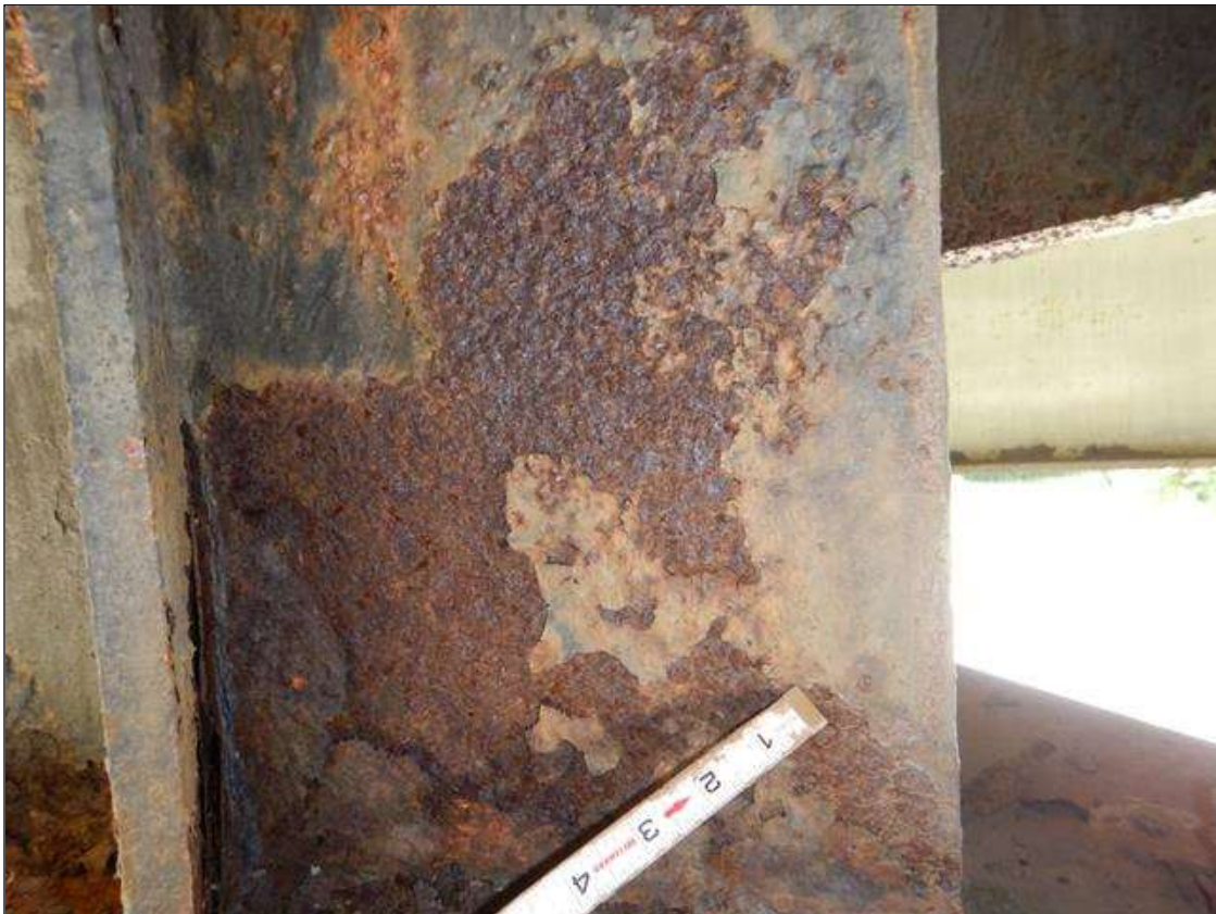
Span 2 Beam 2: At Bent 2, Active Corrosion & Section Loss in lower web, (5/16" Remaining 12" high x 10" long, then 3/8" Remaining 3" high x 12" long,) Bottom Flange (9/16" Remaining full width x 12" long.) (PAR)
