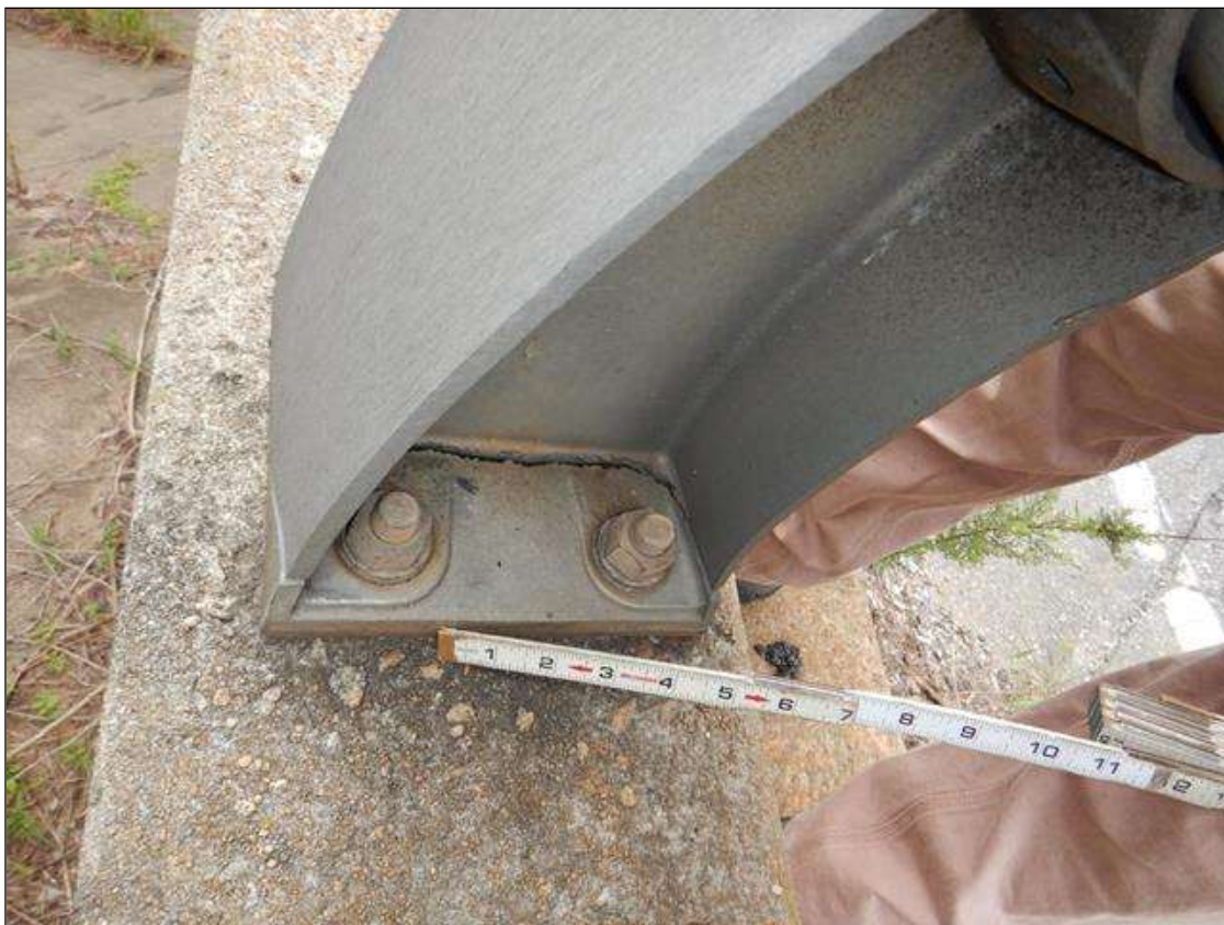
Span 1 Left Bridge Rail: Aluminum Post #1, crack thru web to base plate weld, propagated through flange plates. (PAR)
