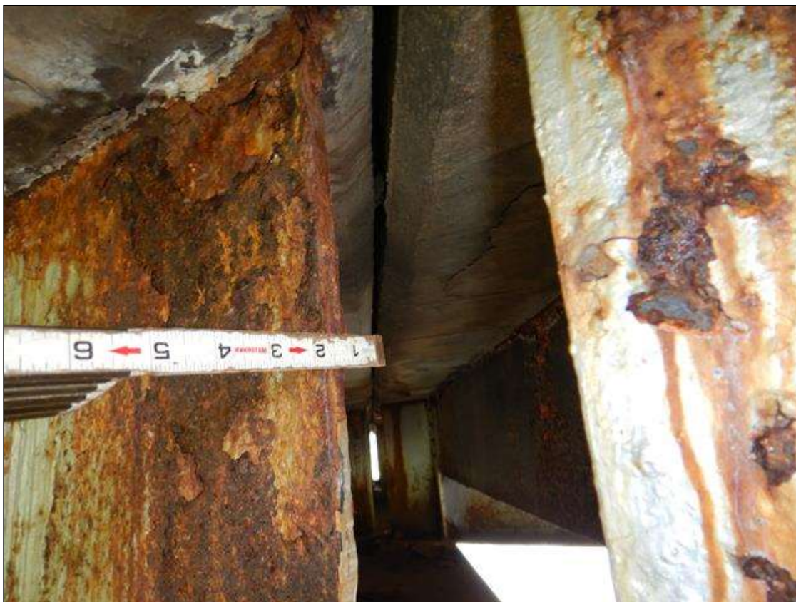
Span 4 Beam 1: BEAM 1, SPAN 4 HAS UP TO 1/8" LOSS ALONG WEB AT PIER 3, 1' HIGH X 1' LONG. (PAR)
