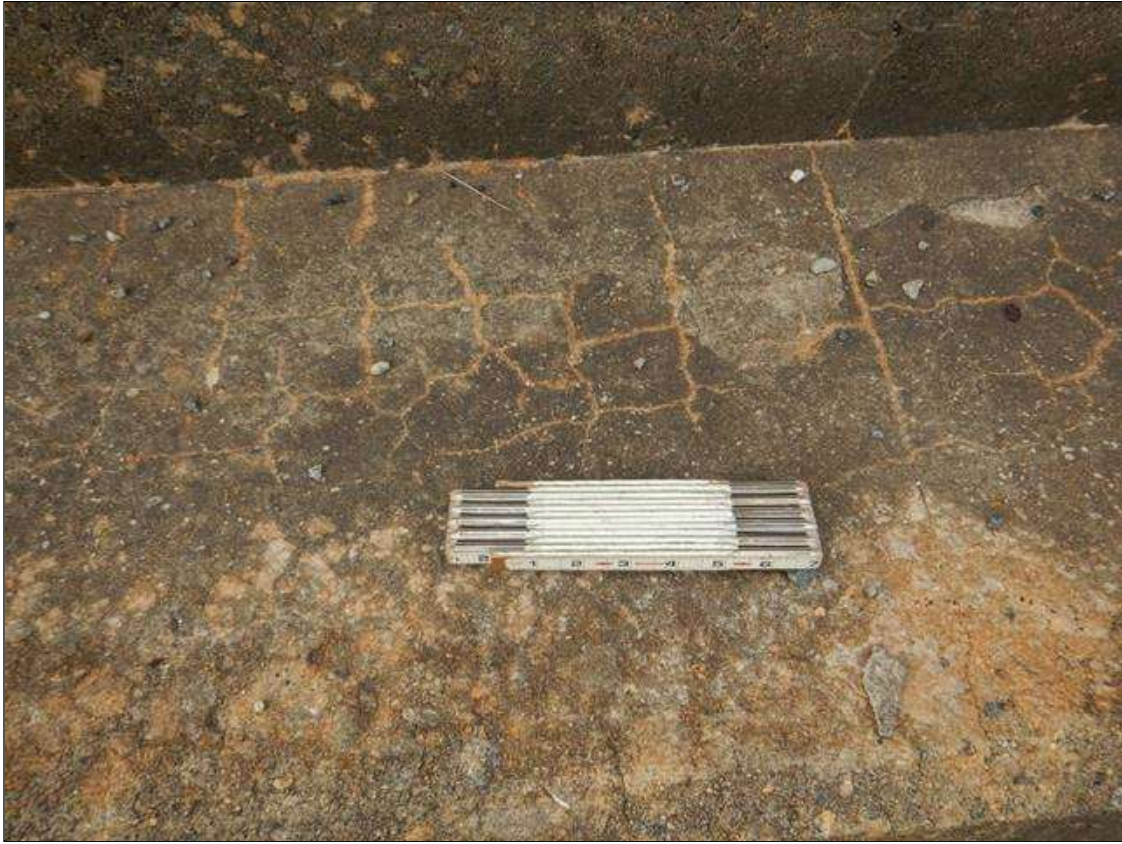
Span 2 Right Bridge Rail: SCATTERED MAP CRACKING ON CONCRETE BASE OF RIGHT BRIDGE RAIL
