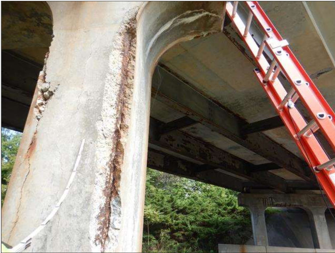
Bent 2 Pile 3: Corner Spalls with Exposed Steel SOUTHWEST FACE (Active Corrosion no measurable Section Loss,) (up to 10' high x 6" x 5",) vertical cracks (1/4" wide x full height) and Delamination in all faces. (PAR)
