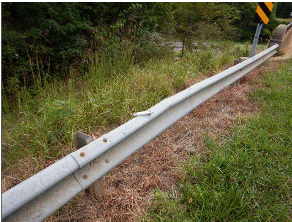
LEFT GUARDRAIL AT WEST APPROACH HAS AREA OF IMPACT DAMAGE FOR 10 FT LONG
