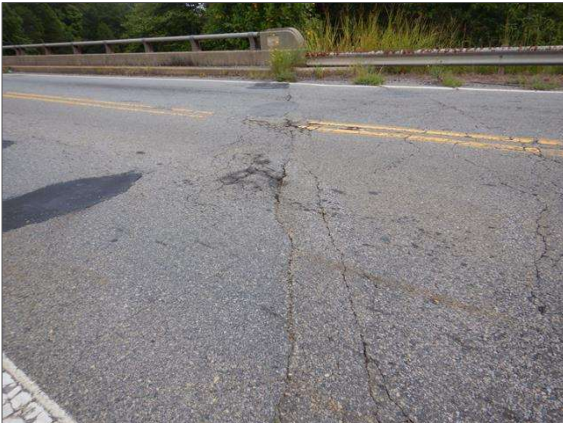
Span 4 Expansion Joint: Top of joint sealed with an Asphalt sealer on wearing surface. CRACKING UP TO 1/4 IN FULL WIDTH WITH PATCHED POTHOLES
