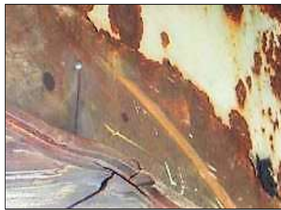
Span 3 Beam 1: NORTH SIDE OF BEAM 1 IN SPAN 3 HAS A 6" LONG X 1/8" WIDE CRACK IN TOP OF BOTTOM FLANGE & EXTENDS INTO WEB ADJACENT TO 10" LONG VERTICAL CRACK IN WEB. (PAR)
