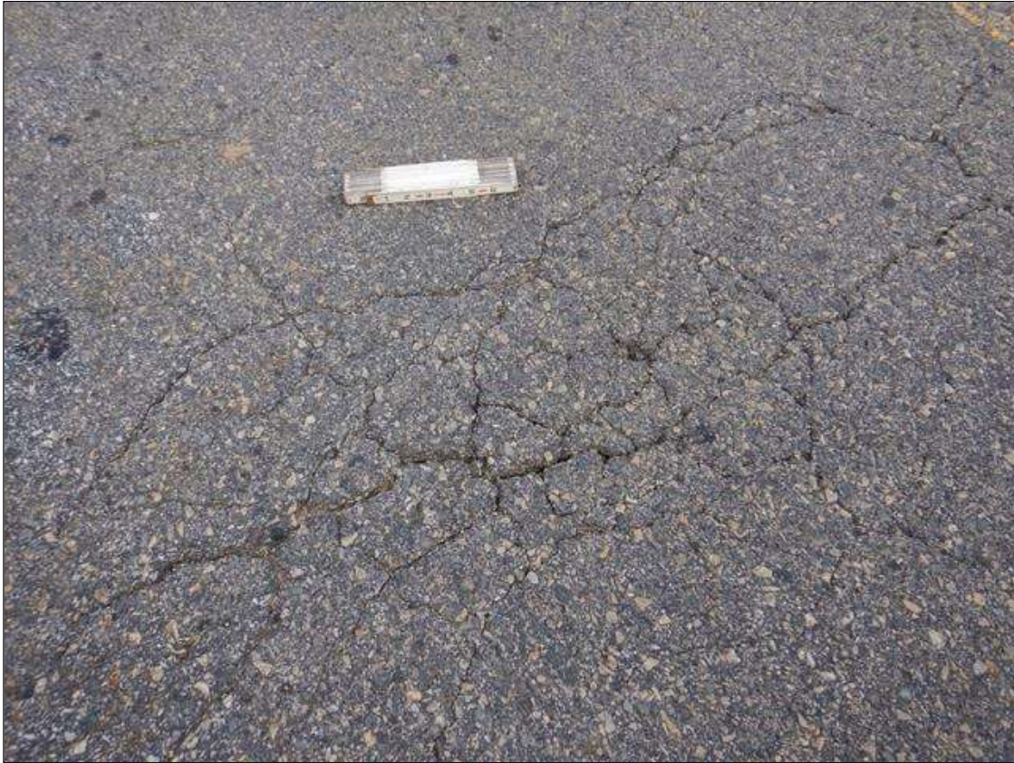
Span 4 Wearing Surface: Map Cracking (up to 1/4" wide) scattered across span in both lanes., SIMILAR CONDITION THROUGH OTHER SPANS IN BOTH TRAVEL LANES
