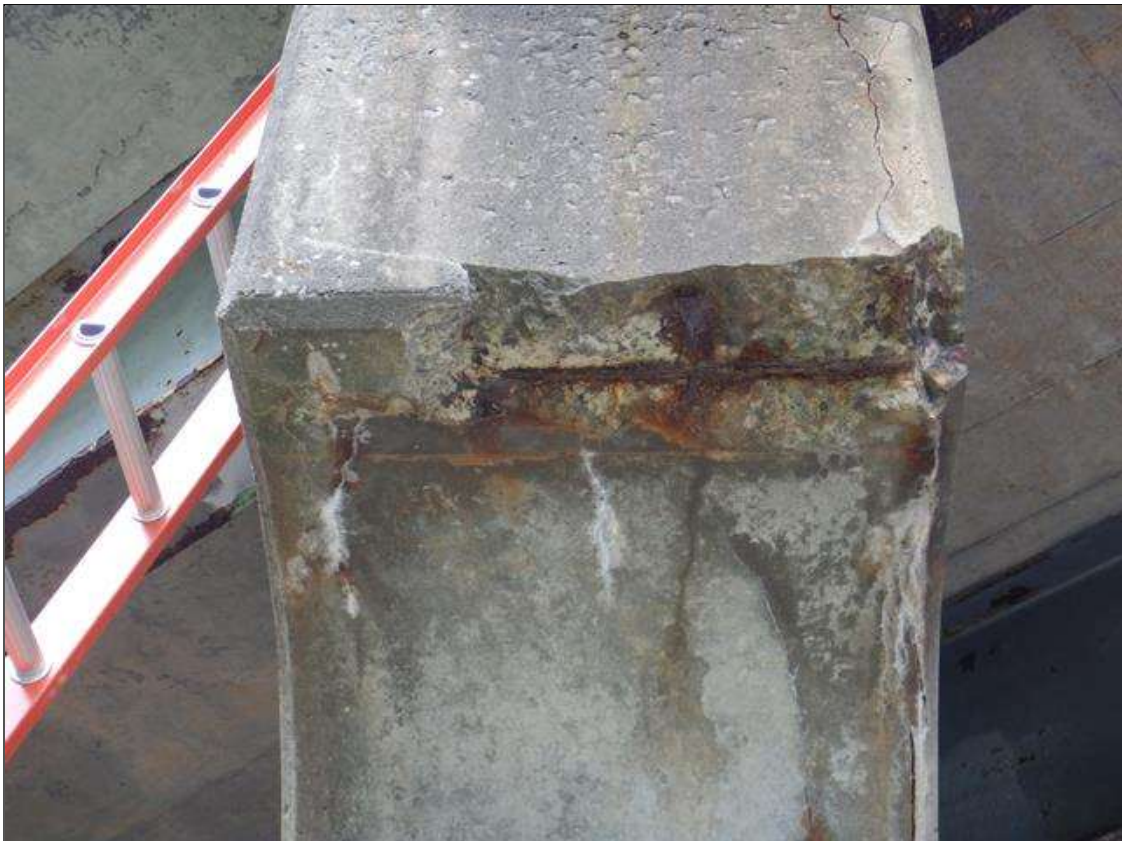
Bent 3 Cap 1: EDGE SPALL AT BEAM AND END CAP ON NORTH END WITH EXPOSED REBAR. 80% SECTION REMAINING IN EXPOSED REBAR. (PAR)
