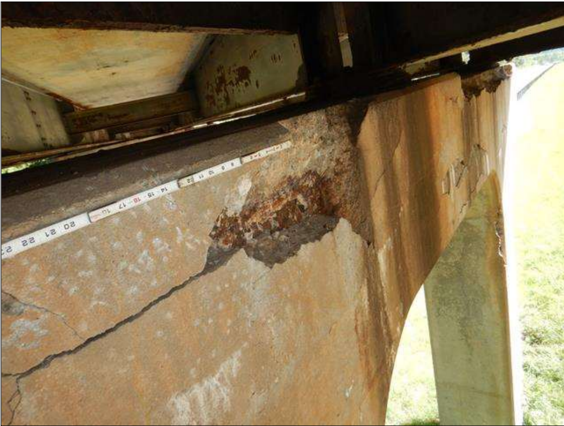
Bent 2 Cap 1: CORNER SPALL IN WEST FACE OF BAY 2 FOR 5 FT WIDE X 1.5 FT HIGH X 4 IN DEEP WITH EXPOSED REBAR. 90% SECTION REMAINING.
