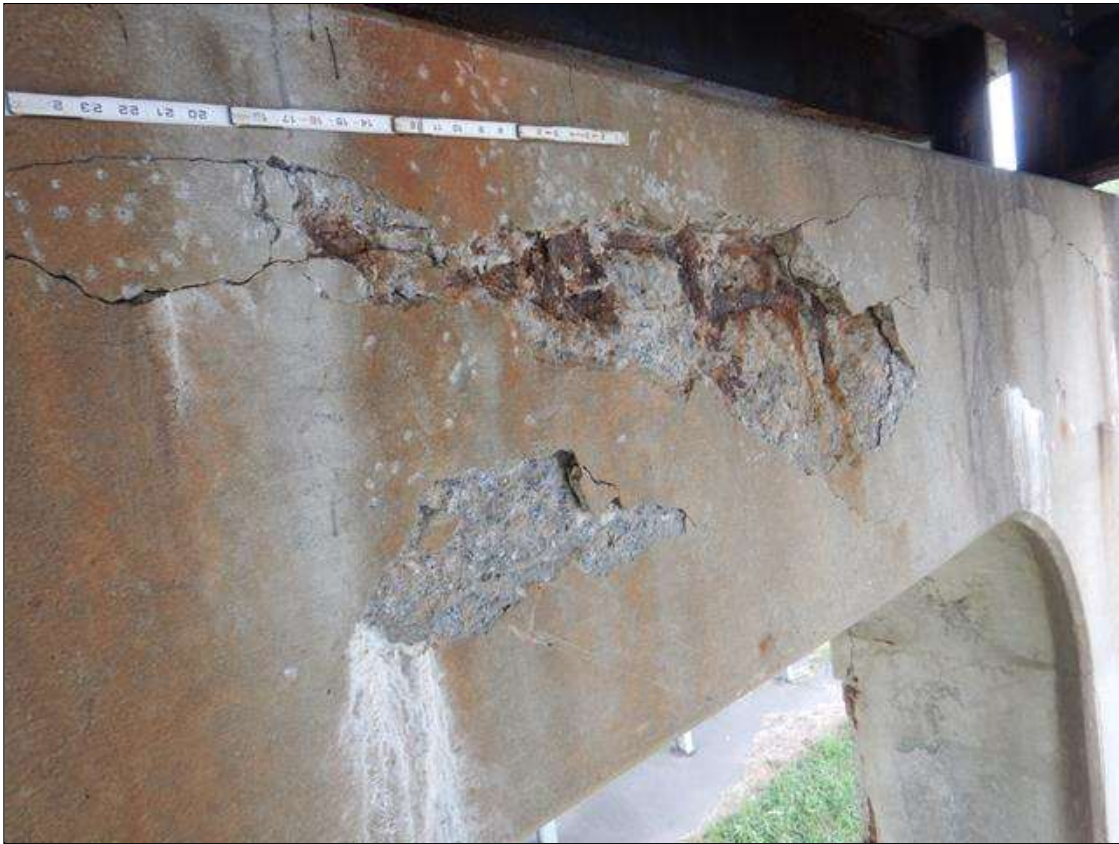
Bent 2 Cap 1: SPALL AT TOP OF CAP IN BAY 1 FOR 5 FT WIDE X 1.5 HIGH X 2.5 IN DEEP WITH 80% SECTION REMAINING IN EXPOSED REBAR EXPOSED REBAR
