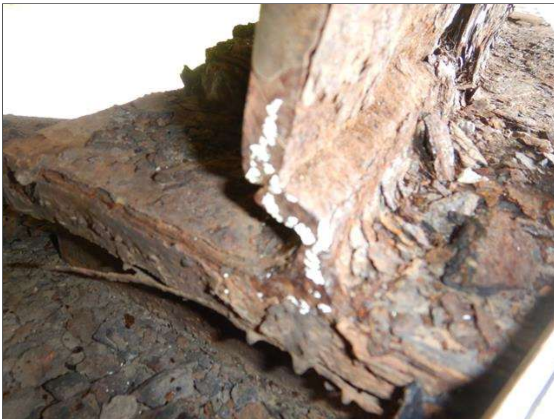
Span 2 Beam 1: DISTORTION FOR 9 IN LONG X 1 IN HIGH AT BOTTOM OF WEB INSIDE OF WEB IS CRACKED. HOLE IN WEB 3 IN IN DIAMETER 9 IN FROM FAR BEARING. (PAR)
