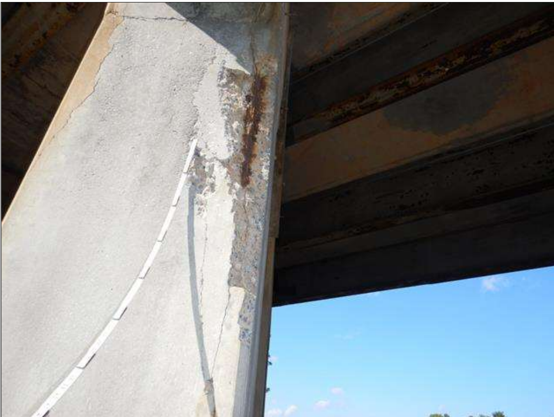
Bent 1 Pile 3: Southeast Corner, near cap, Spall with Exposed Steel (Active Corrosion no measurable Section Loss), vertical cracking 1/8" wide and Delamination (5' high x 1' x 1'.) (PAR)
