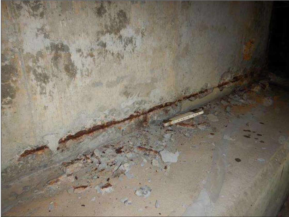
End Bent 2 Abutment: DELAMINATED SPALLED AREA IN BOTTOM CENTER OF BACKWALL IN BAY 1 NEXT TO BEAM 2 FOR 6 FT LONG X 4 IN HIGH X 1/2 IN DEEP WITH EXPOSED REBAR. 80% SECTION REMAINING IN EXPOSED REBAR
