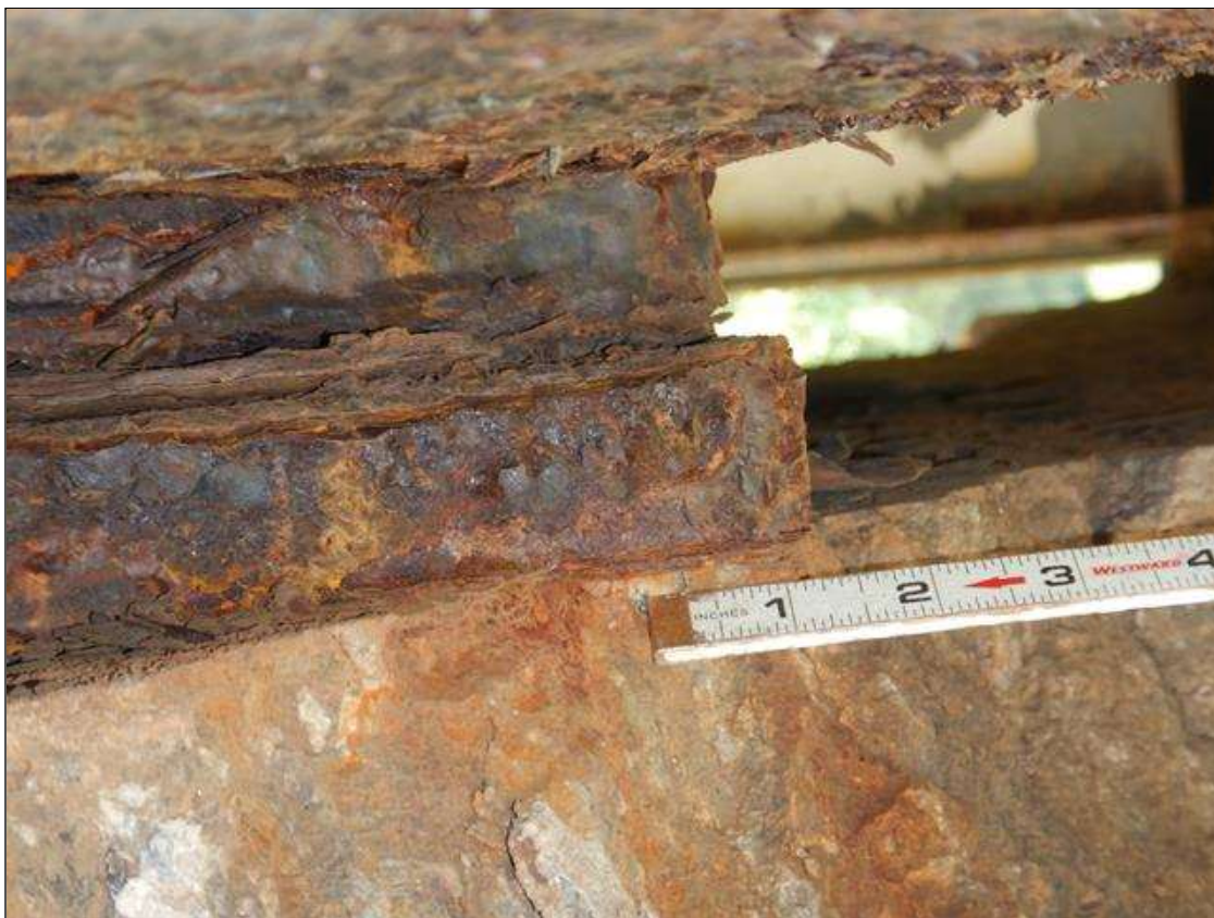
Span 3 Near Bearing: 1 IN UNDERMINING ON BEARING PLATE DUE TO SPALL. (PAR)
