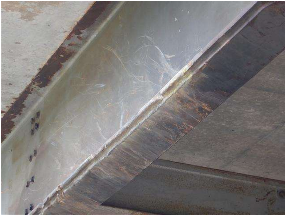
Span 3 Beam 4: Impact damage due to high loads, with Out of plane bending in bottom flange and web. Numerous Points of impact located approximately between 12' and 30' from Bent 3, above US220 North bound lanes. See NCDOT Special Inspections Damage Report dated 21 November, 2011
