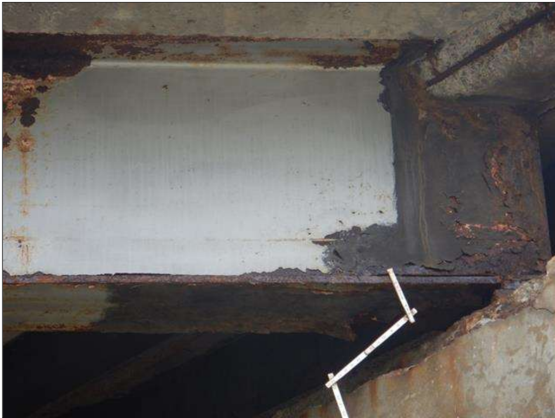
Span 2 Beam 4: at Bent 2, beginning 12" from beam end, Active Corrosion & Section Loss in lower web, (1/2" Remaining 3" high x 4' long,) Bottom Flange (3/4" Remaining 5" wide x 4' long.) (PAR)
