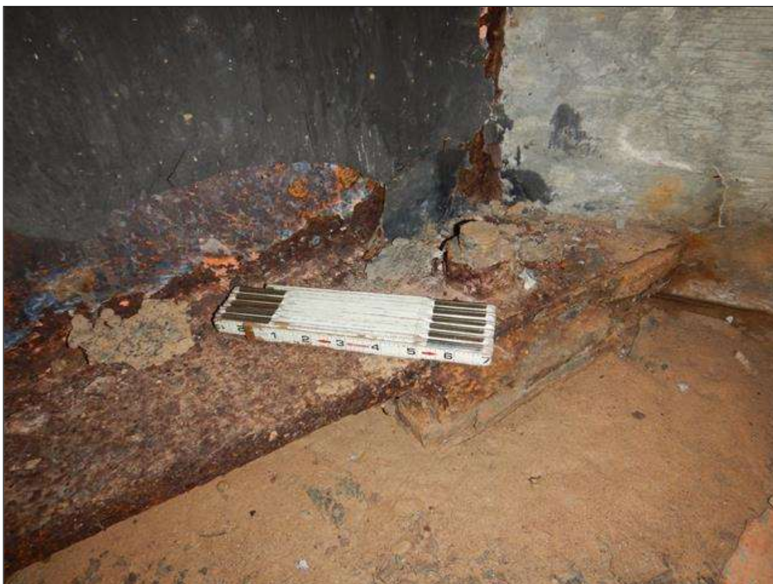
Span 1 Beam 4: at End Bent 1, Rust and Scale no measurable Section Loss in bottom flange and lower web.
