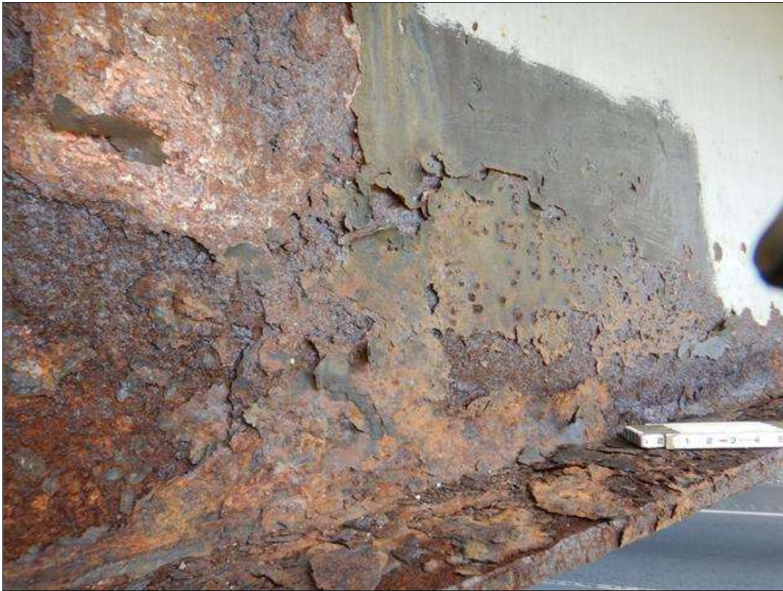
Span 3 Beam 4: at Bent 2, Active Corrosion & Section Loss in Web (5/16" Remaining 9" high x 15" long,) Bottom Flange (11/16" Remaining full width x 15" long.) (PAR)
