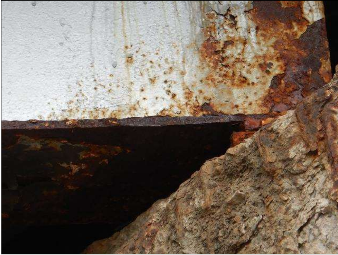
Span 3 Beam 4: at Bent 3, Active Corrosion & Section Loss in lower web, (3/8" Remaining 8" to 4" high x 30" long,) Bottom flange, (9/16" Remaining full width x 18" long,) (Previous PAR 2021 INSPECTION VERIFIED VISUALLY, LADDER ACCESS UNSAFE.) (PAR)
