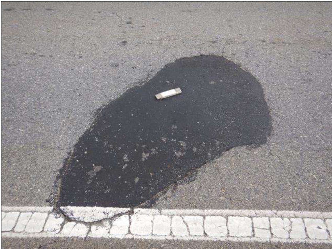
Span 4 Wearing Surface: BOTH LANES OF TRAVEL HAVE SEVERAL SCATTERED PATCHED AREAS THAT ARE SOUND, PERIMETER OF PATCHES ARE DELAMINATED
