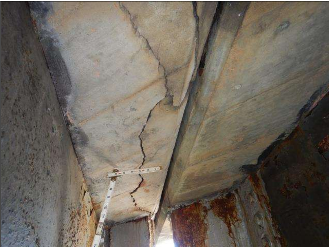
Span 1 Deck: UNDERSIDE DECK HAS CRACKING UP 1/4 IN WIDE X FULL WIDTH IN BAYS 1-3. BAY 1 PICTURED
