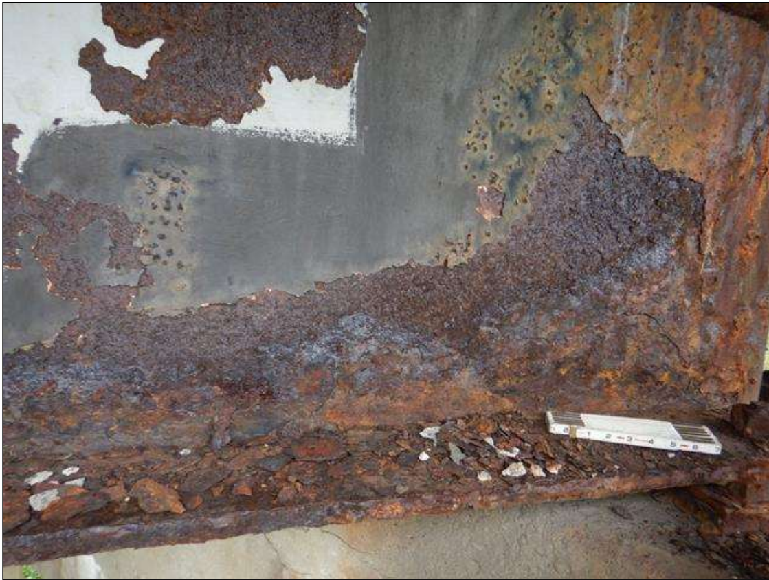
Span 3 Beam 1: at Bent 2, Active Corrosion & Section Loss in lower web, (3/8" Remaining 4" high x 4' long,) Upper Web (3/8" Remaining 5" high x 17" long,) Bottom Flange (3/4" Remaining full width x 3' long.) (PAR)
