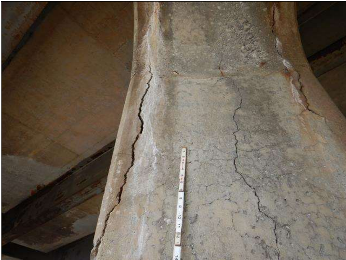
Bent 3 Pile 2: Vertical cracks (1/4" wide) with rust staining and Delamination (imminent spalling) West face, (8' high x 2' wide.) (PAR)
