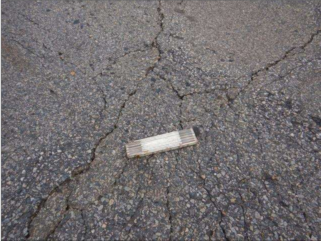
EAST APPROACH HAS MAP CRACKING UP TO 1/4 IN WIDE WITH SOME AREAS OF SUNKEN PAVEMENT
