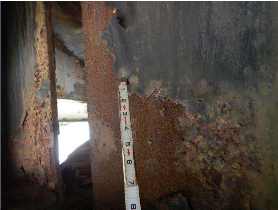
Span 3 Beam 3: at Bent 2, Active Corrosion & Section Loss in Lower Web (5/16" Remaining 12" high x 10" long, then 3" high x 12" long,) Bottom Flange (9/16" Remaining full width x 2' long.) (PAR)
