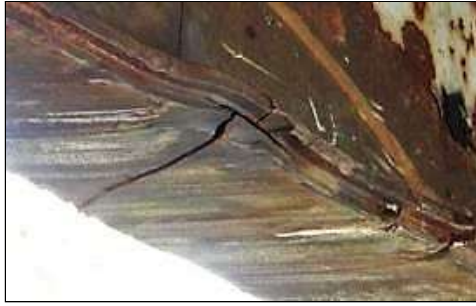
Span 3 Beam 1: 10 1/2" LONG X 3/16" WIDE CRACK IN BOTTOM FLANGE COVER PLATE TO BEAM 1 IN SPAN 3 , LOCATED 23 FT FROM BENT 3 BEARING. (PAR)
