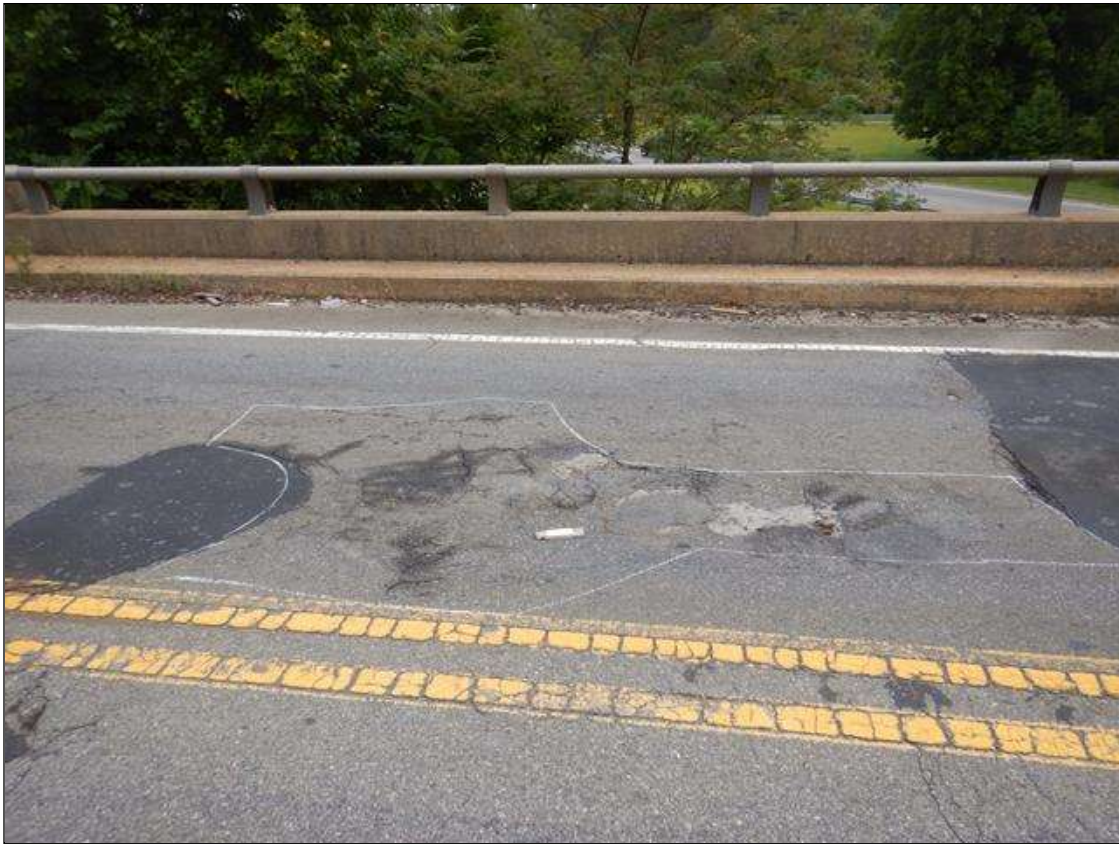
Span 1 Wearing Surface: LEFT TRAVEL LANE AT BEGIN OF SPAN 1 HAS DELAMINATED SPALLED AREA FOR 14 FT LONG X 6 FT WIDE X UP TO 1 IN DEEP
