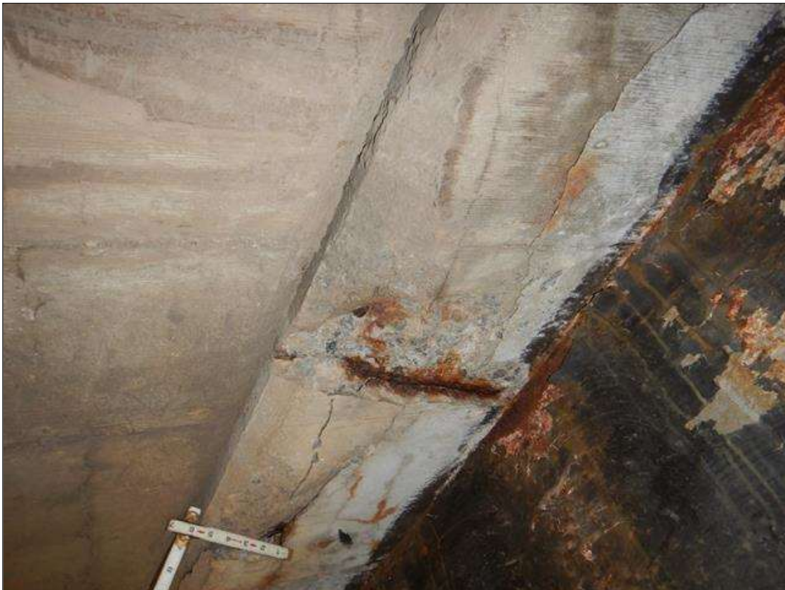
Span 3 Deck: DELAMINATION WITH SPALL FOR 1 FT LONG X 6 IN WIDE X 2 IN DEEP WITH EXPOSED REBAR IN DECK UNDERSIDE AT BENT 3 IN BAY 2 NEXT TO BEAM 2
