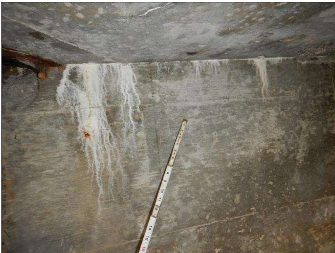
End Bent 1 Abutment: AREAS OF EFFLORESCENCE AT TOP OF BACK WALL IN BAY 3
