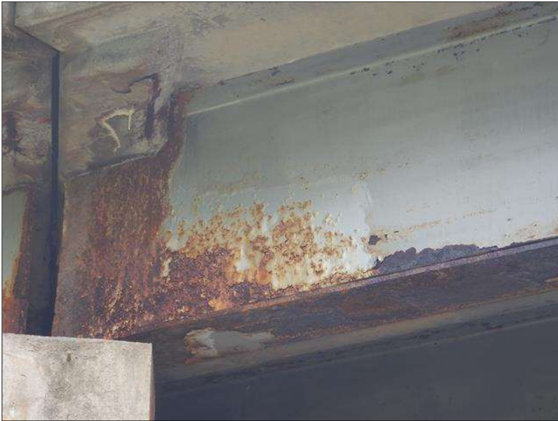
Span 2 Beam 4: at Bent 1, Active Corrosion & Section Loss in Web (down to 3/8" Remaining full height x 12"), Bottom Flange (9/16" to 3/4" Remaining full width x 12" long.) (PREVIOUS PAR VISUALLY INSPECTED DUE TO UNSAFE ROAD CONDITIONS FOR LADDER SETUP)
