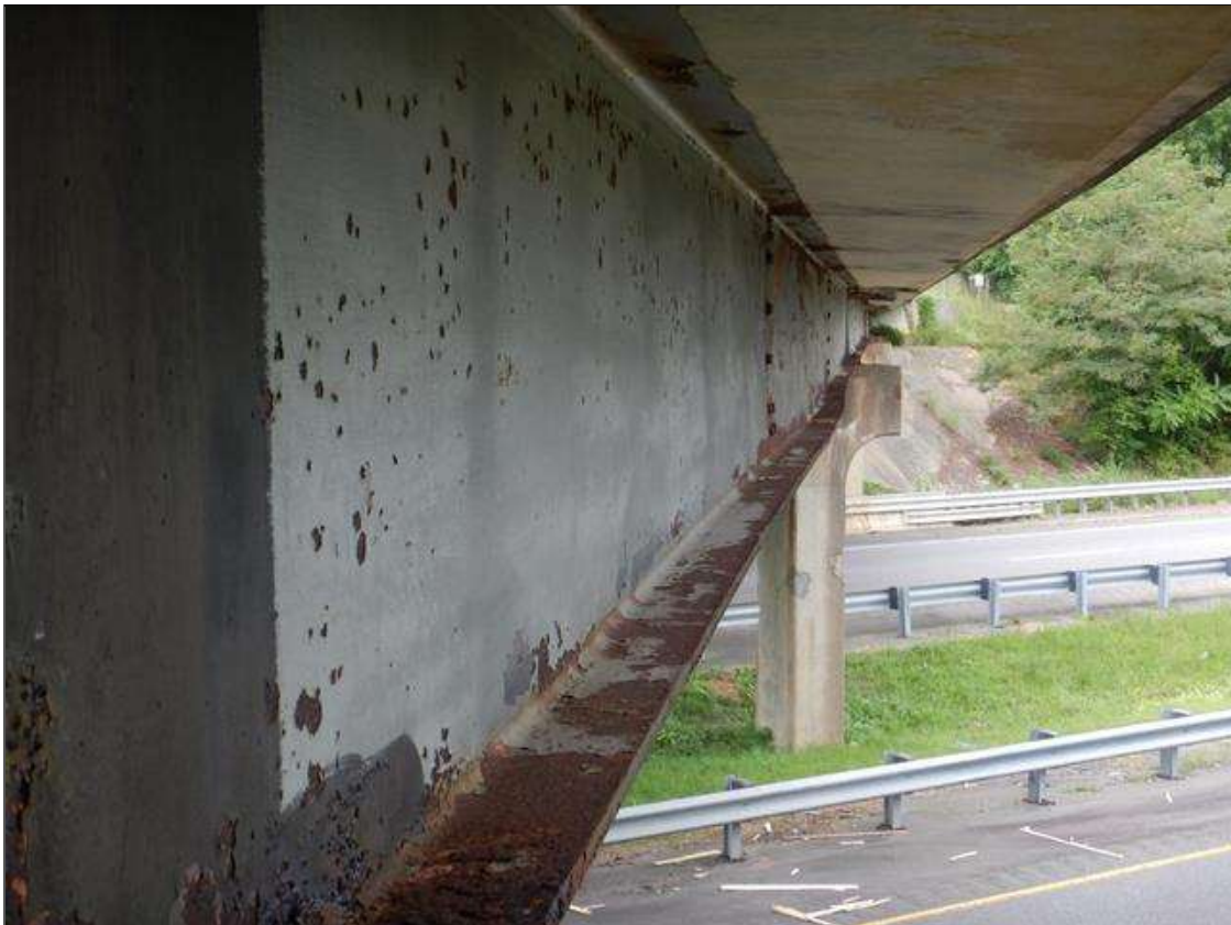
Span 3 Beam 1: Impact damage due to high load, with Out of plane bending in bottom flange and web. Point of impact located approximately 18' from Bent 3, above US220 North.
