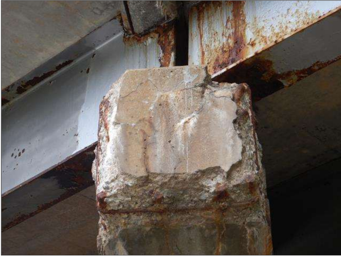
Bent 3 Cap 1: EDGE SPALL AT BEAM AND END CAP ON NORTH END FOR 2 FT LONG X 1 FT WIDE X 2 IN DEEP, WITH EXPOSED REBAR. 80% SECTION REMAINING IN EXPOSED REBAR. (PAR)
