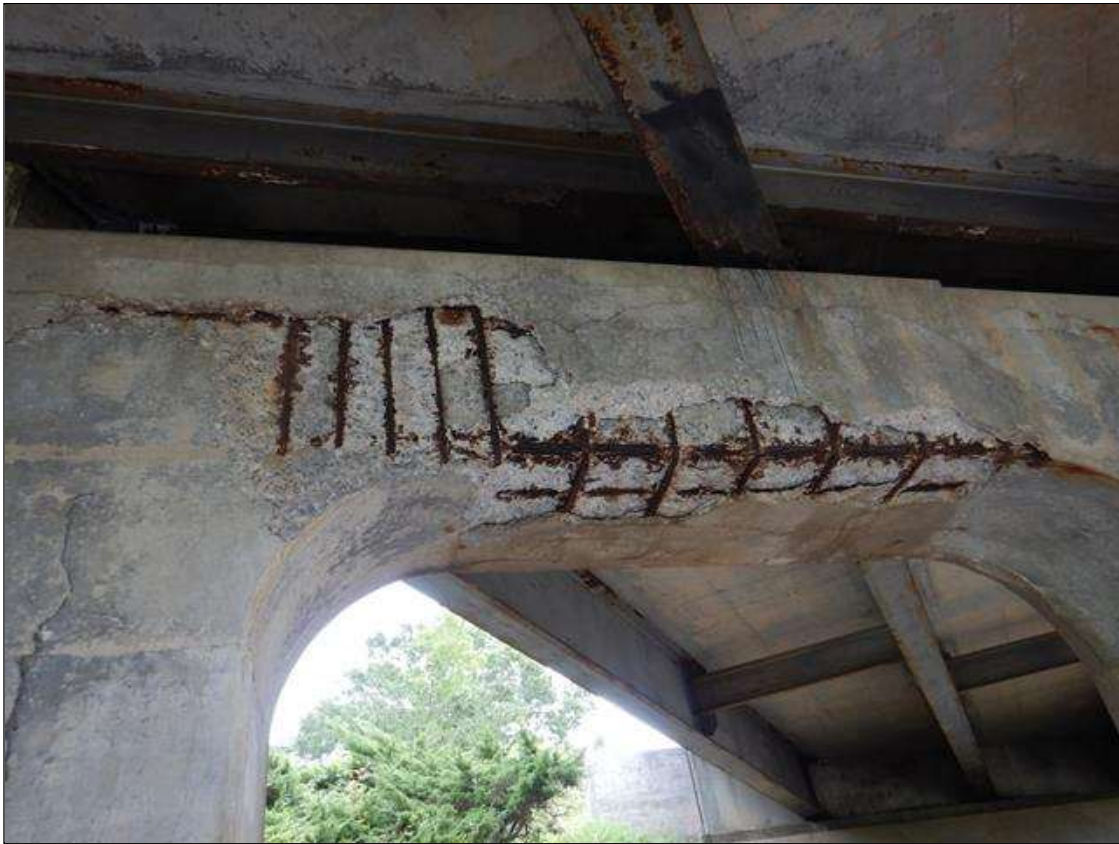
Bent 3 Cap 1: from beam 4 to north end, Top, bottom, east, west and north faces, Spalling with Exposed Steel (up to 4" deep) (Active Corrosion no measurable Section Loss), Cracks (1/4" wide) with rust stains and efflorescence, and Delamination 30' long x up to full height x up to full width.) Spalling/ Delamination on Top corners up to 6" wide, No Bearing Loss for beams 1, 2, or 3. (PAR.)
