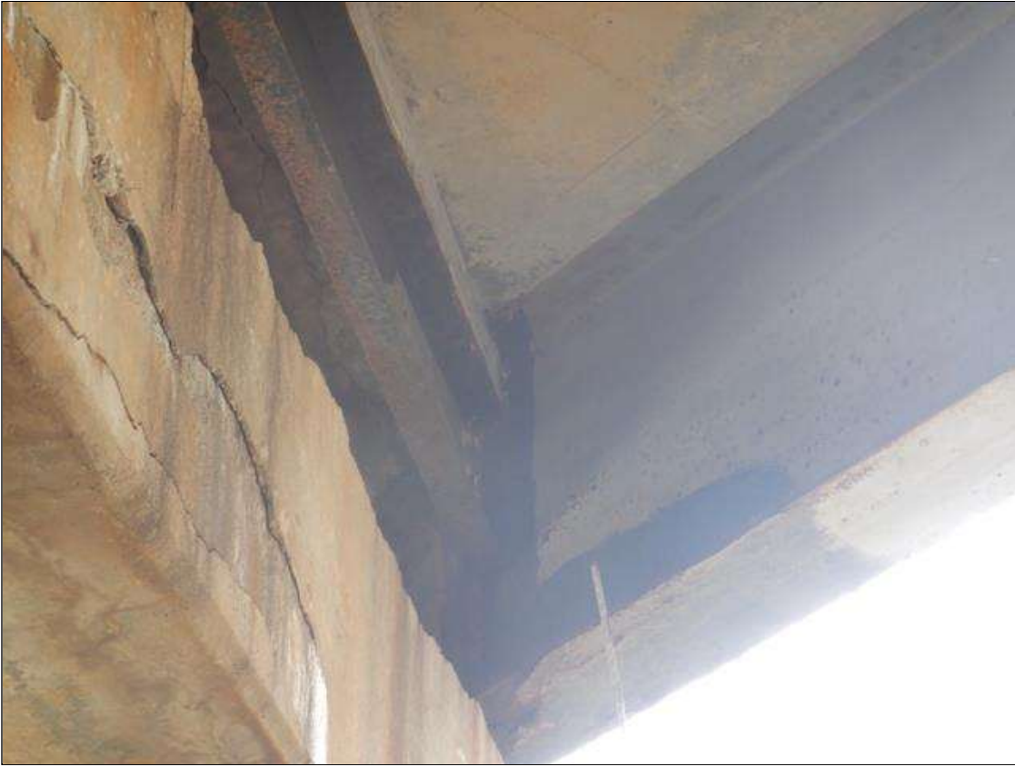
Span 2 Beam 4: at Bent 2, Active Corrosion & Section Loss in Bottom flange in front of bearing (5/8" Remaining full width x 12" long,) lower web, (5/16" Remaining 12" high x 10" long,) Upper Web (5/16" Remaining 12" high x 10" long,) Web stiffener / diaph connection plate (5/8" Remaining 5" x 4".) (PREVIOUS PAR VISUALLY INSPECTED DUE TO UNSAFE ROAD CONDITIONS FOR LADDER SETUP)
