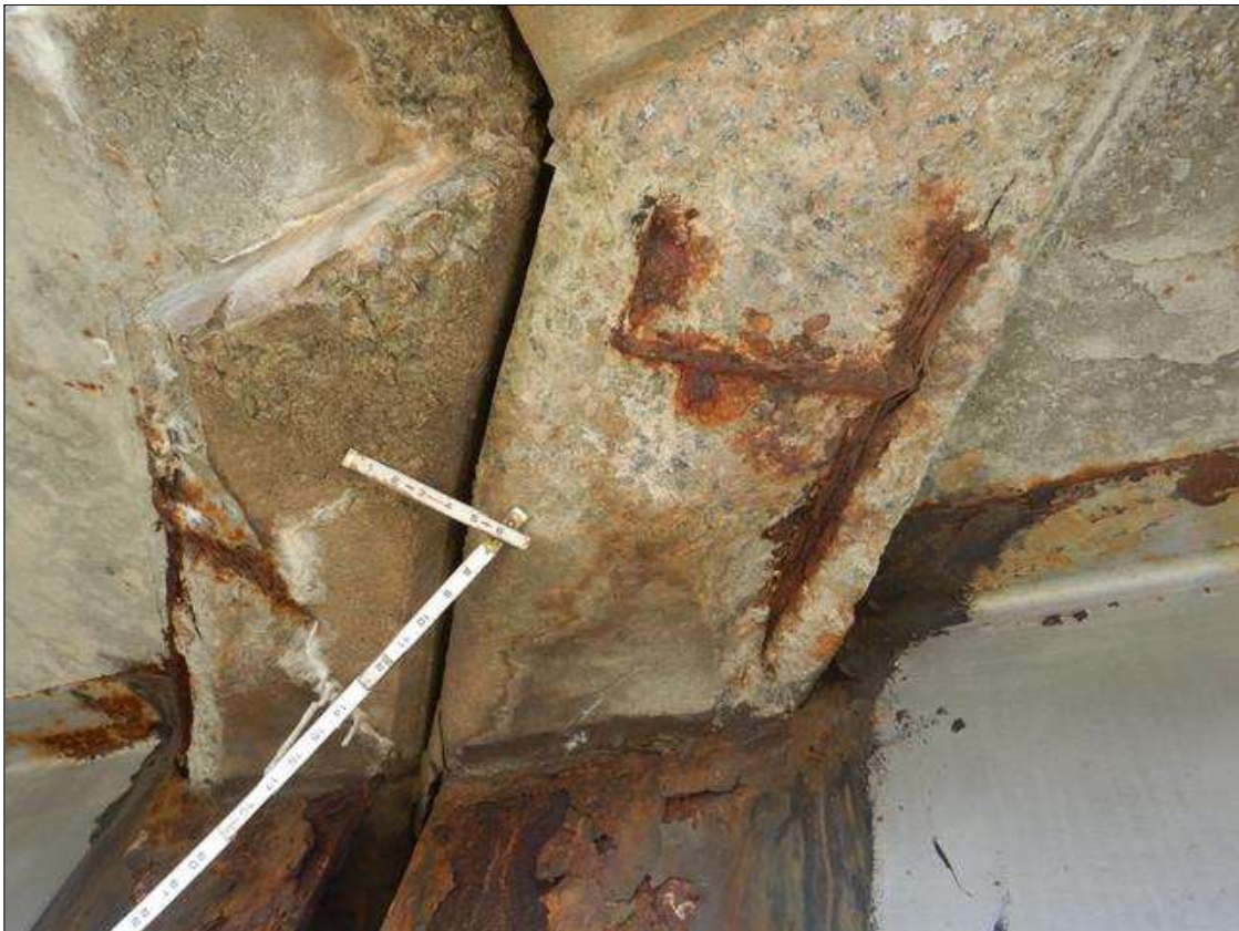
Span 2 Beam 4: RC end diaphragm at Bent 1, right overhang, Cracks (1/8" wide) and Delamination/ Spall with Exposed Steel (24" x 1 FT x 4" deep.) 80% SECTION REMAINING ON EXPOSED REBAR
