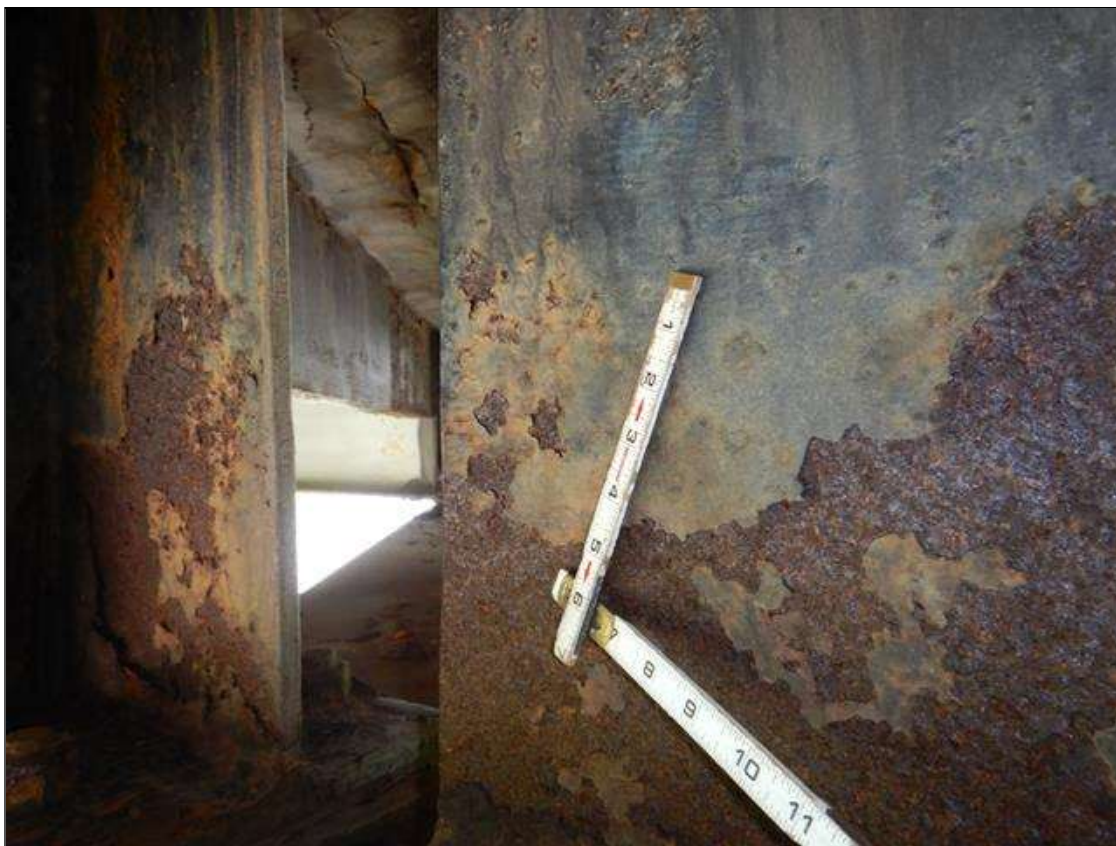
Span 3 Beam 2: at Bent 2, Active Corrosion & Section Loss in lower web, (3/8" Remaining 8" high x 12" long,) Bottom flange, Rust and Scale no Section Loss. (PAR)
