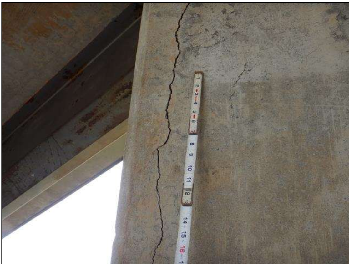
Bent 3 Pile 1: near cap, Northwest Corner, vertical cracks (1/4" wide x 3' long) with Delamination (6" x 4" x 3'.)
