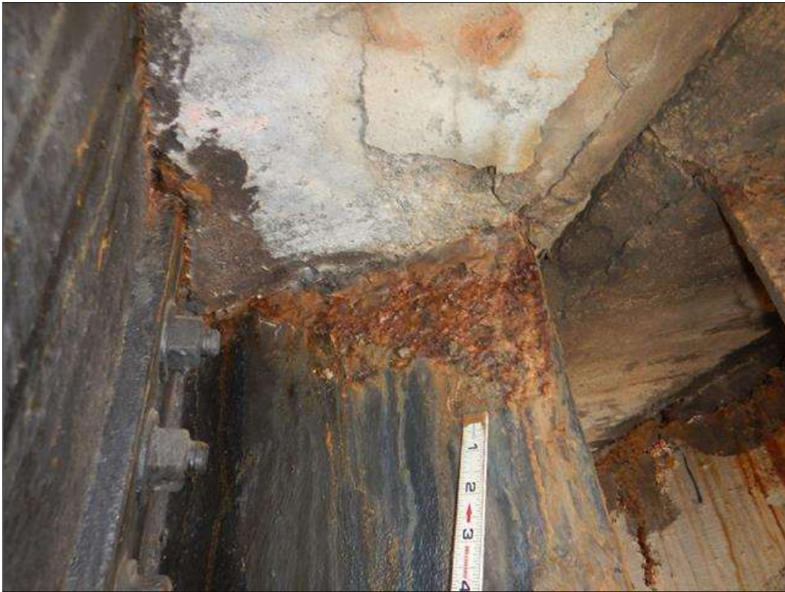
Bent 2 Cap 1: Top corners of cap, east and west faces, in bay 3 to south end, Spall with Exposed Steel (Active Corrosion no measurable Section Loss) and Delamination 6' long x up to 12" high x up to 10" wide.). (PAR)
