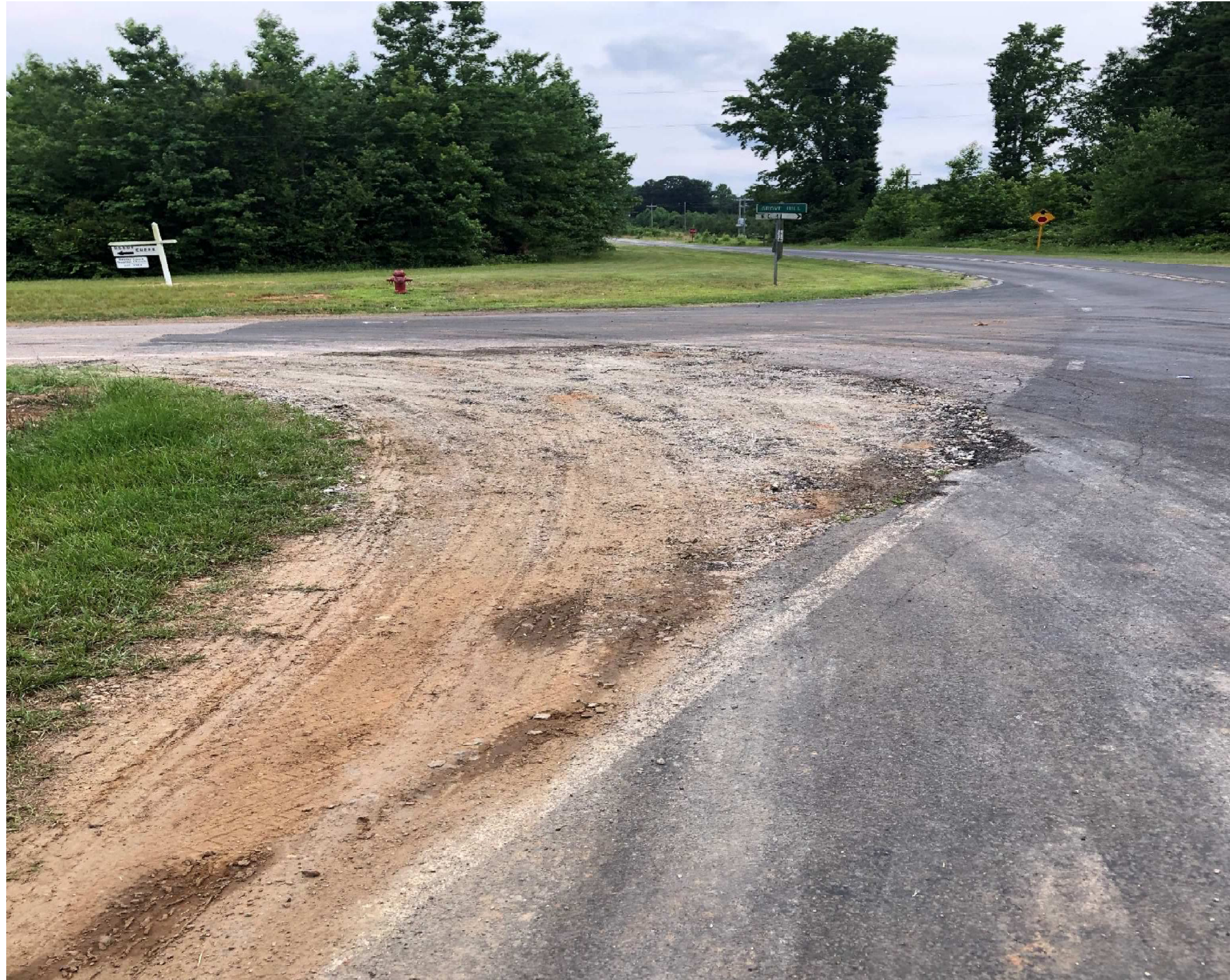
Map 7 - Widen the radius at the northeast corner of the intersection of SR 1510 – Hardy Cemetery Rd and SR 1512 – Reedy Creek Rd. with 5.5" of B25.0C and 1.5 " of S9.5B.
