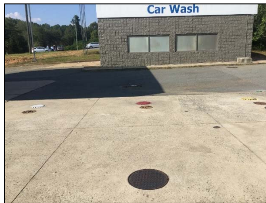
Fuel USTs, with car wash
