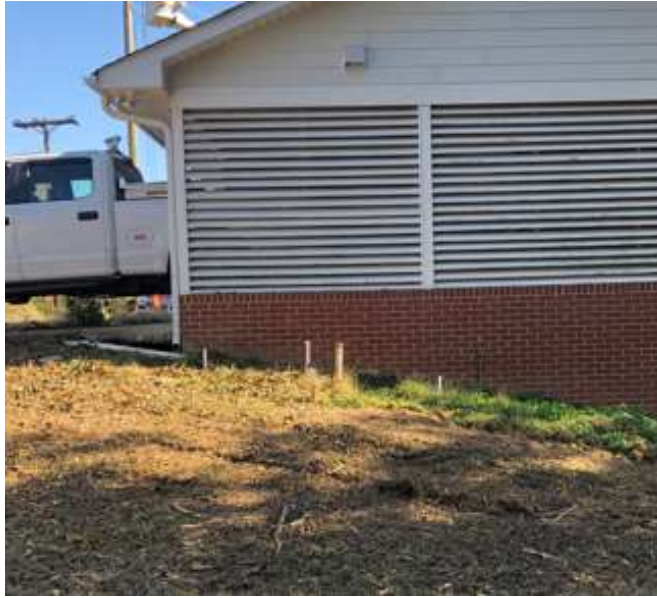
Heating Oil UST located adjacent to the west facing exterior wall of the single-family residential structure (11.16.2021)
