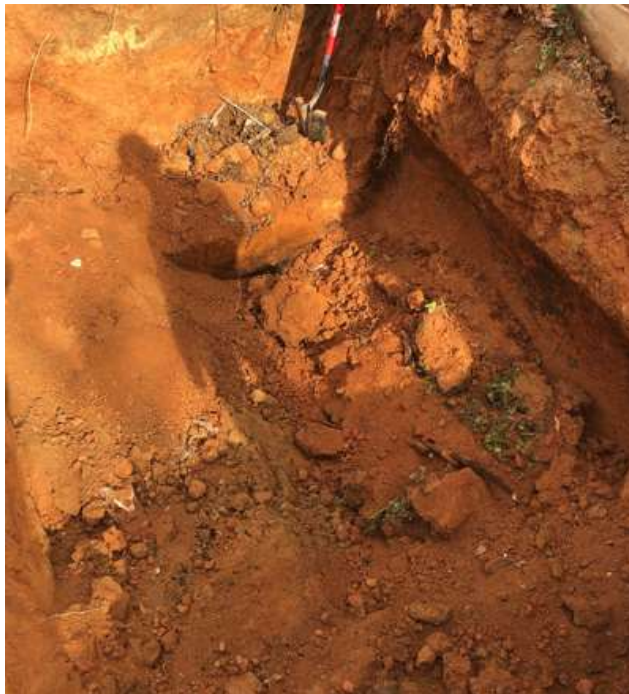
Tank grave upon removal (12.01.2021)
