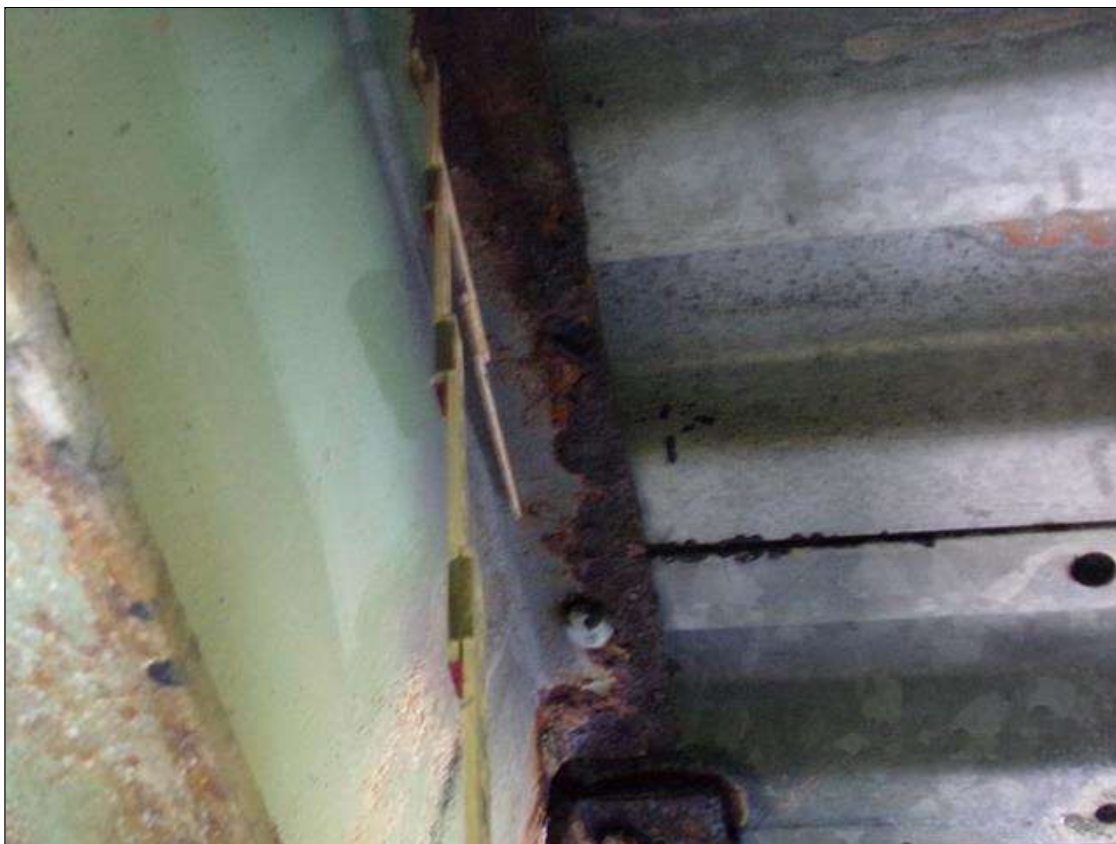
Span 3 Beam 7: 18" x 2" area of 1/8" section loss (3/8" remaining) on both sides of top flange at Bent 2 (PAR)
