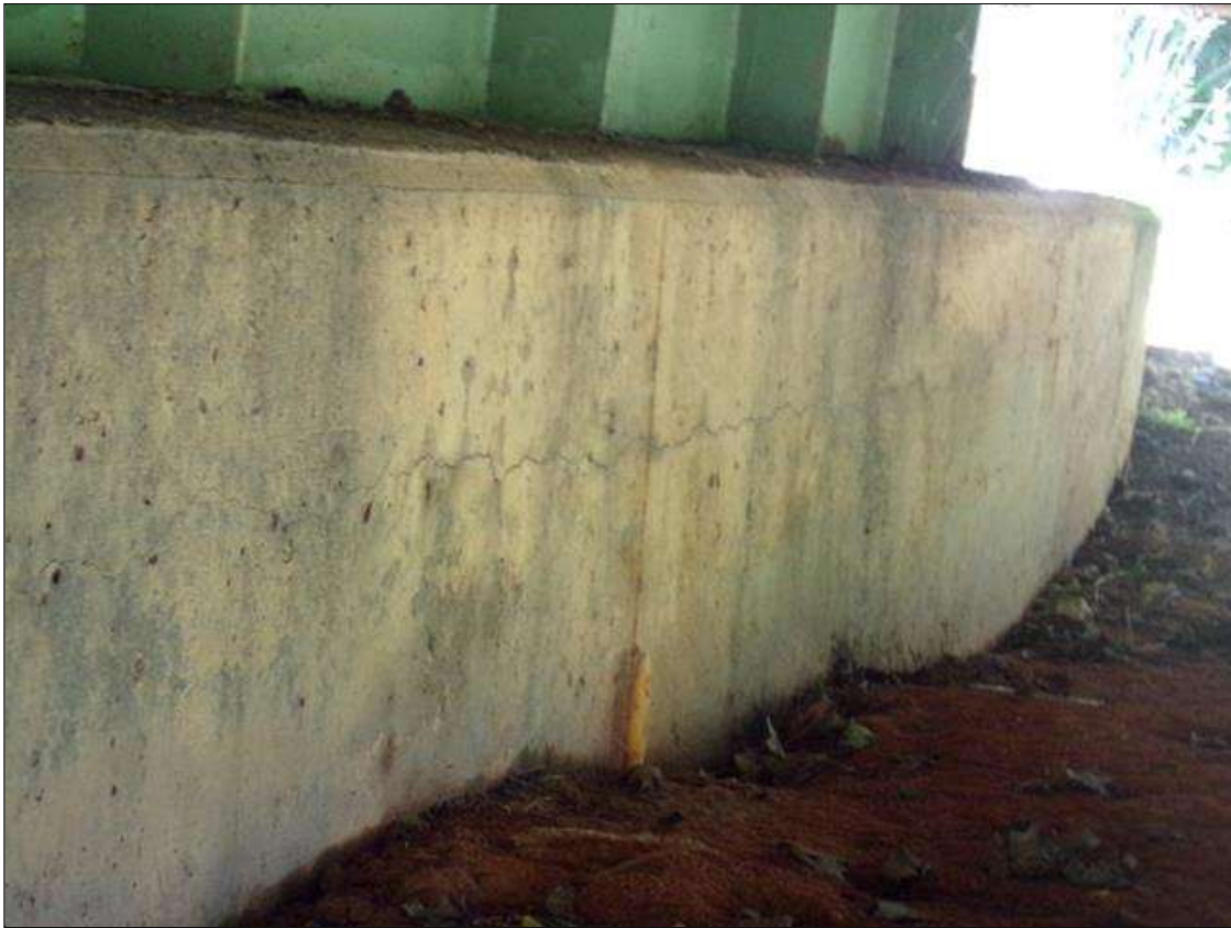
End Bent 1 Abutment: 24' x UP TO 1/16" HORIZONTAL CRACK THROUGHOUT EAST FACE OF ABUTMENT BETWEEN BEAMS 2 THROUGH 10. (PHOTO TAKEN BETWEEN BEAMS 3 AND 4)
