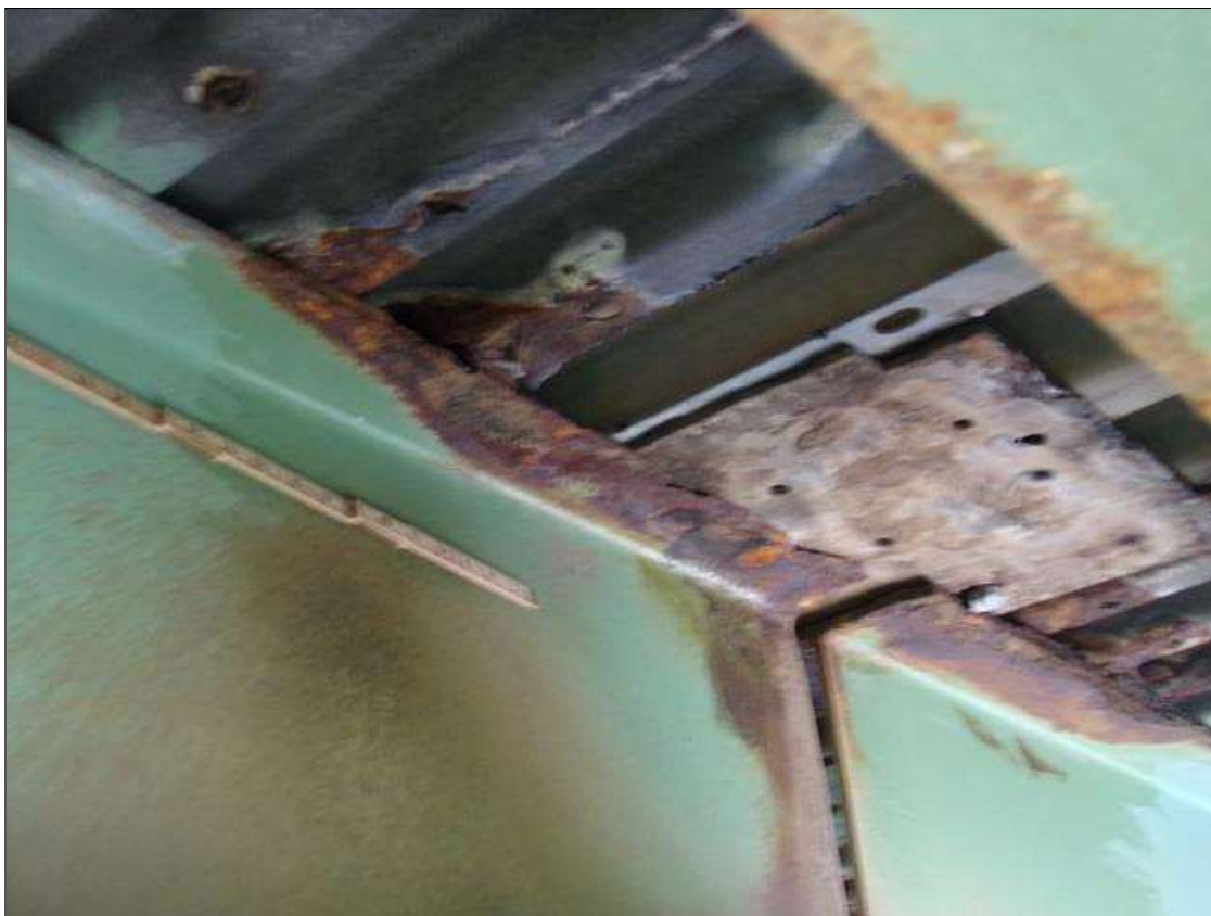
Span 1 Beam 5: 20" x 3 1/2" area of section loss (with knife edge remaining) on right side of top flange at Bent 1 (PAR)
