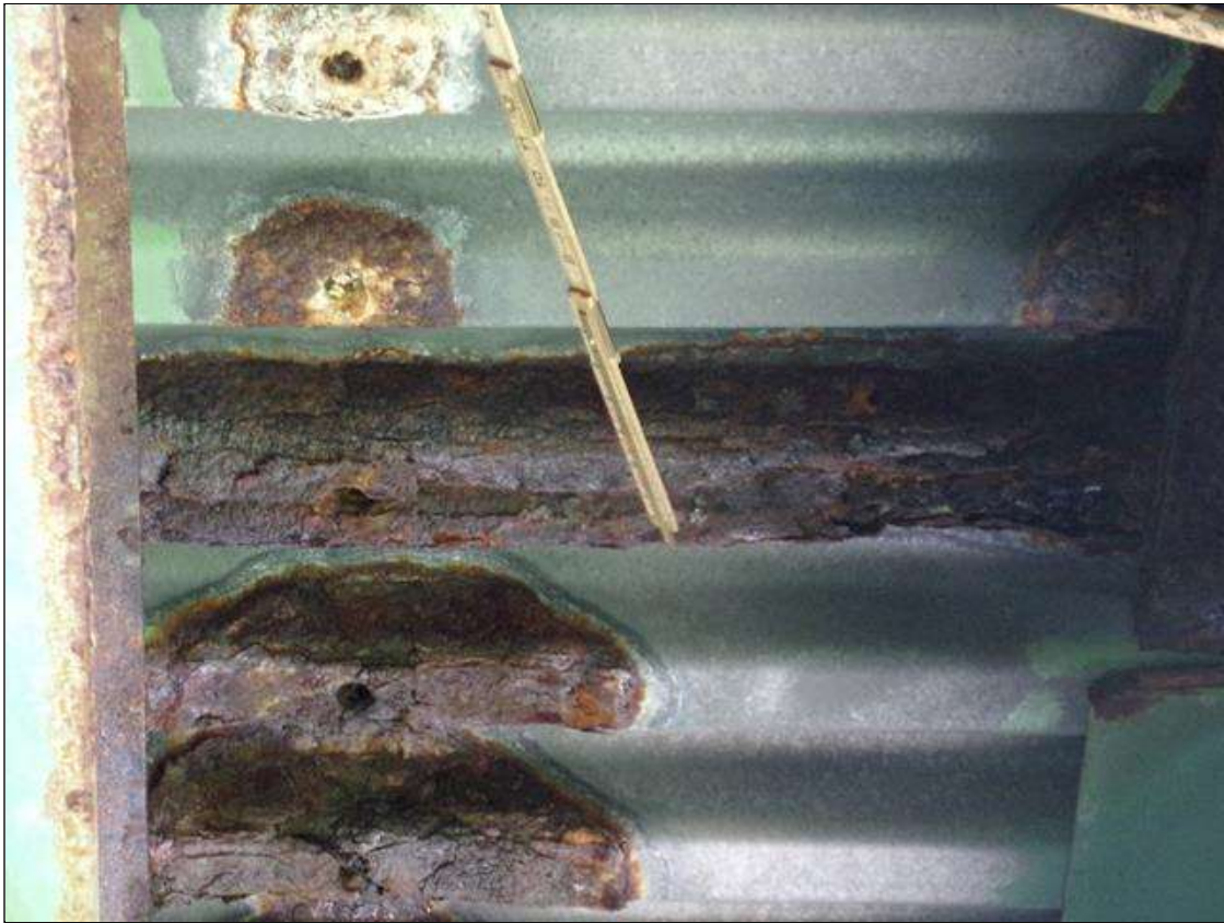
Span 1 Deck: 1/2 SF RUST SCALE WITH 100% LOSS OF SECTION AND CONCRETE DECK EXPOSED BETWEEN BEAMS 8 AND 9 AT BENT 1. (PAR)
