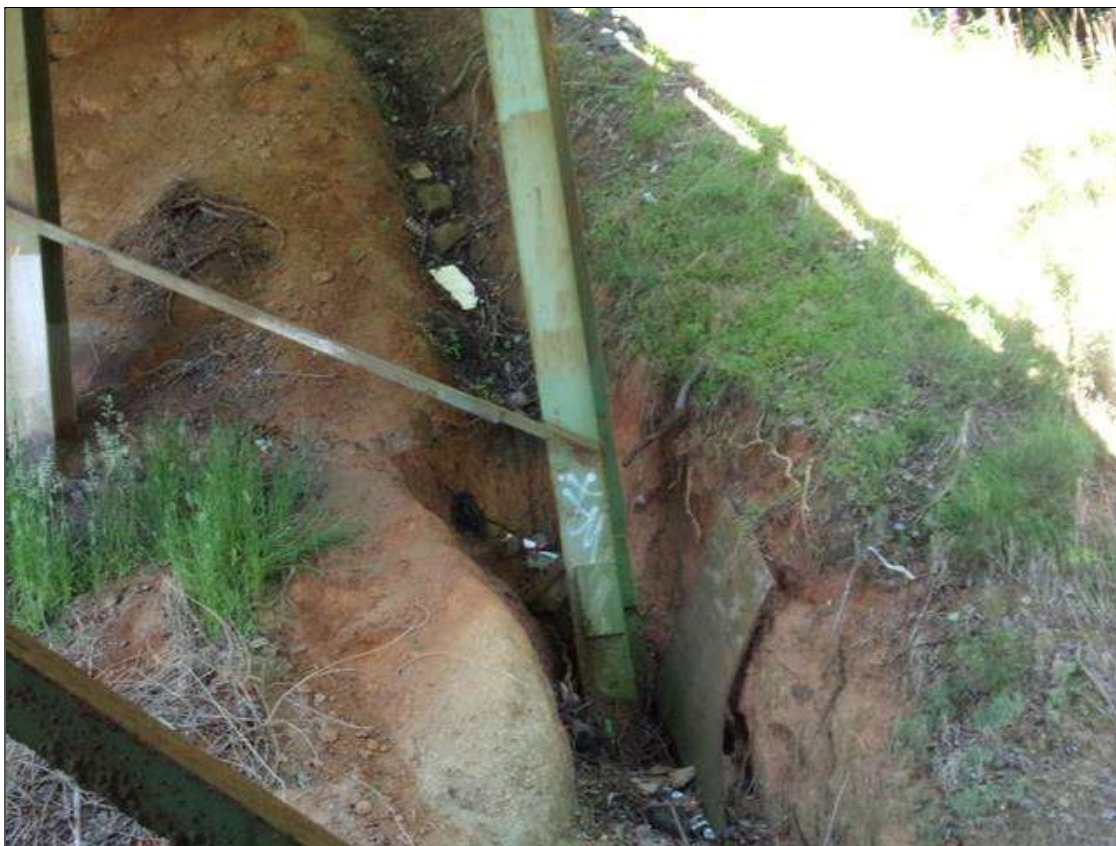
Bent 1 Pile 1: 20' x 7' x 6' deep erosion on End Bent 1 slope
