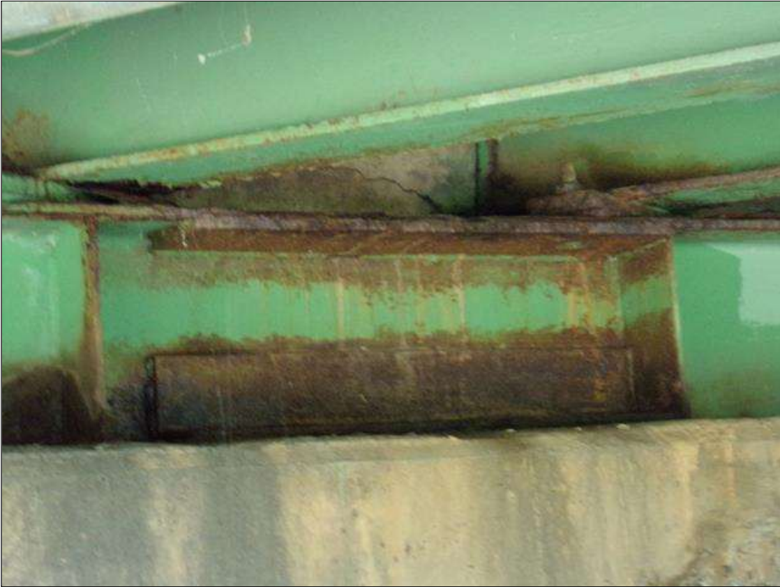
END BENT 1 CAP: 1/4" WELDED PLATE REPAIR TO TOP FLANGE WITH ADDED ANGLE PLATES TO THE BOTTOM FLANGE AND WEB BETWEEN BEAMS 6 AND 7.
