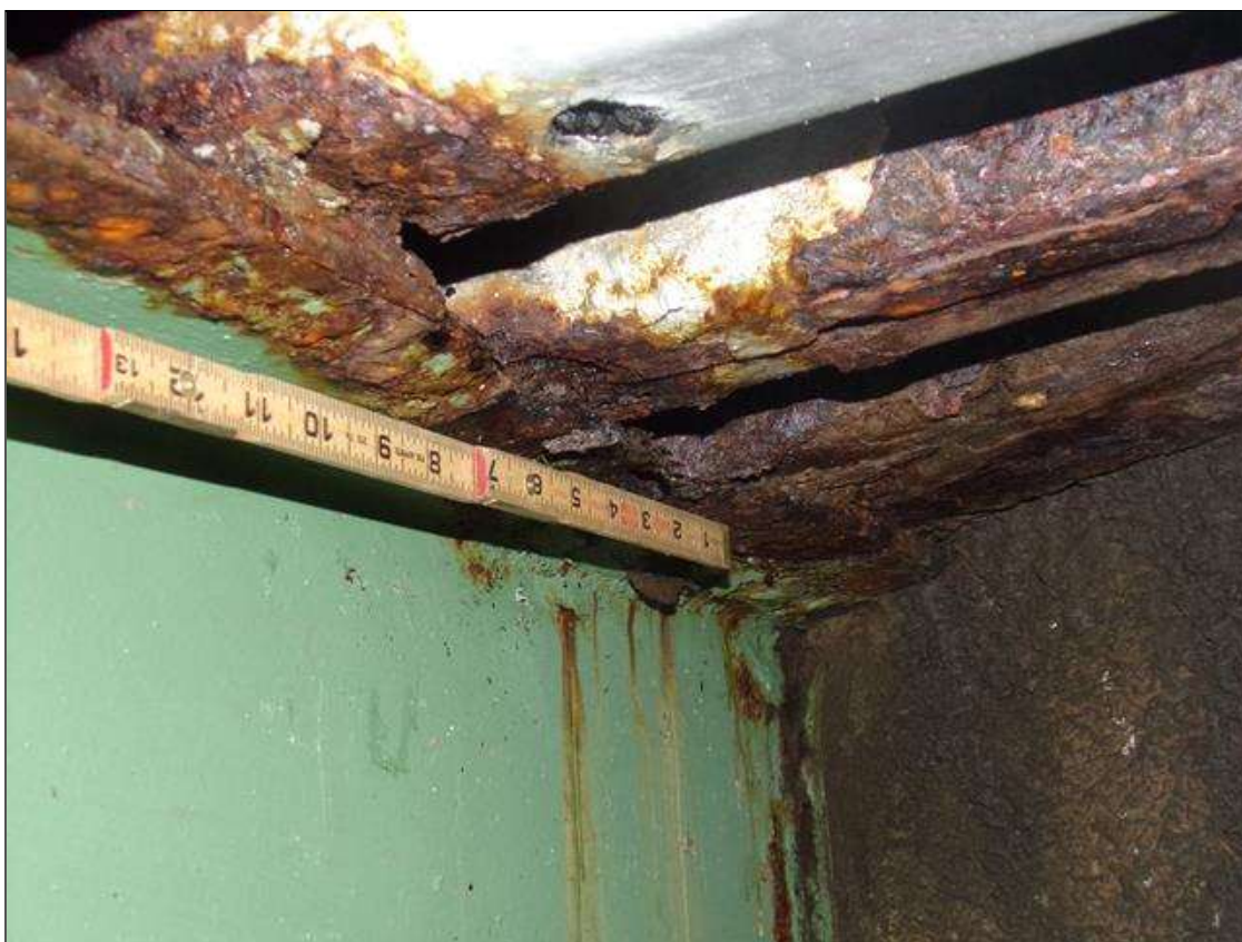
Span 3 Beam 7: 32" RUST SCALE TOP FLANGE WITH SECTION LOSS TO KNIFE'S EDGE AND 9" x 1" area of 100% section loss ON BOTH TOP FLANGES AT END BENT 2. (PAR)
