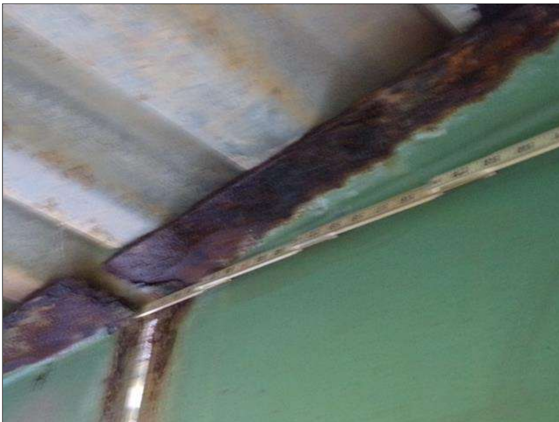
Span 1 Beam 7: 14" x 3" area of 1/4" section loss (1/4" remaining) on both sides of top flange at Bent 1 (PAR)
