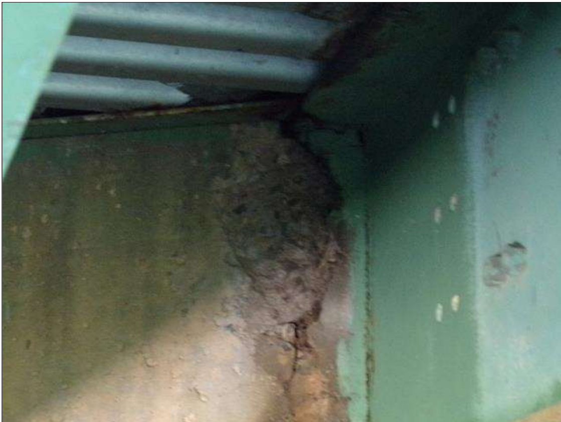
End Bent 2 Abutment: (5) UP TO 9" x 21" x 1 1/2" SPALLS and area of delamination ON NORTH BEAM INTERFACE IN ABUTMENT BACKWALL AT BEAM ENDS BETWEEN BEAMS 8 THROUGH 12.
