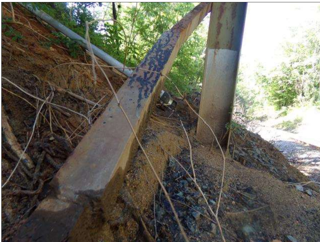
BENT 2 PILE 1: 3' ANGLE PLATE WELDED REPAIR TO CROSS BRACING MEMBER ON EAST FACE AT MID Span.
