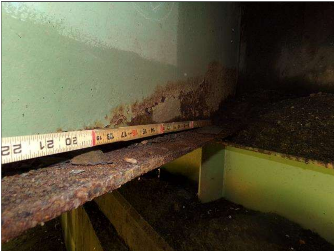
Span 3 Beam 6: 4' RUST SCALE BOTTOM FLANGE UP TO 8" IN WEB WITH 1/4" REMAINING IN BOTTOM FLANGE AT END BENT 2. (PAR)
