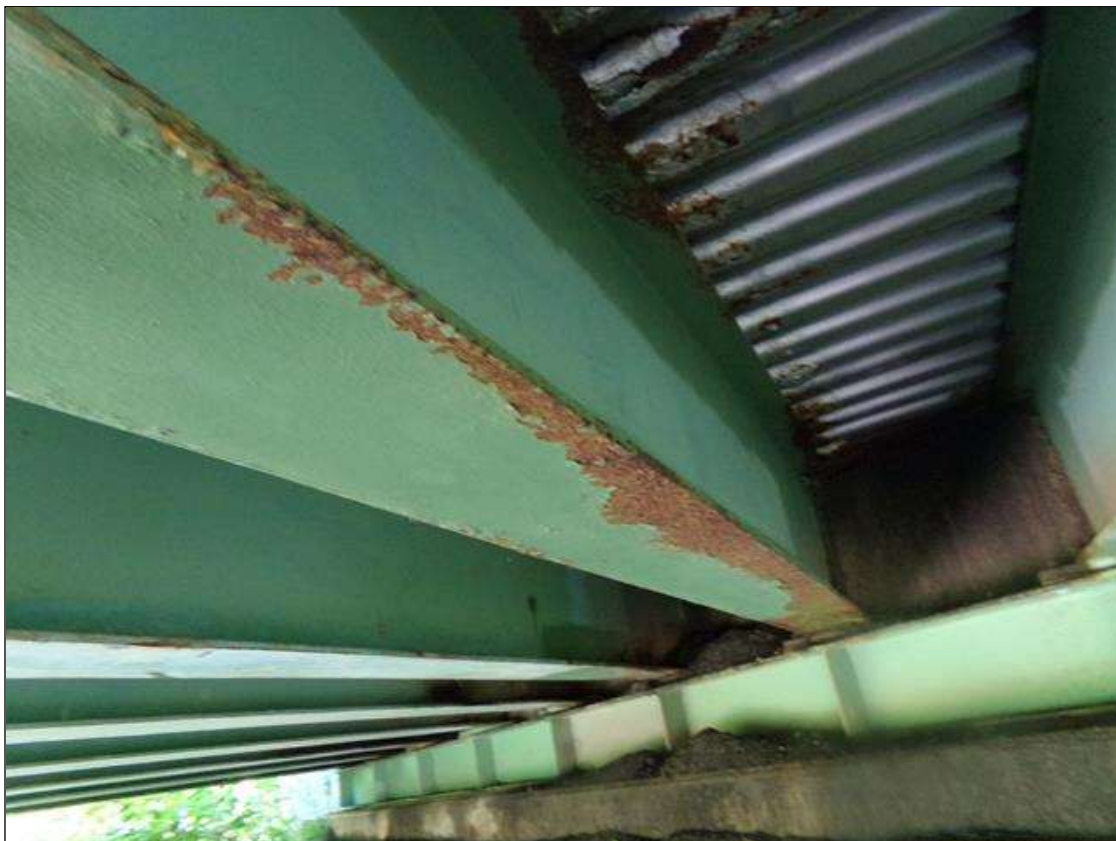
Span 3 Beam 7: 20' peeling paint with rust
