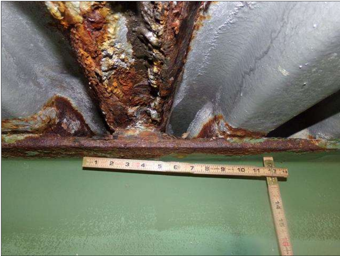
Span 3 Beam 7: 15" x 1" area of 1/8" section loss (3/8" remaining) on left side of top flange, 6' from End Bent 2 (PAR)
