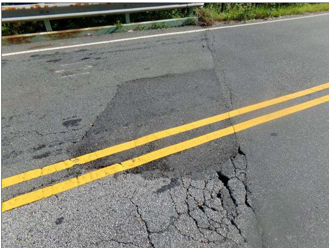
Span 3 Wearing Surface: (2) UP TO 5' x 3' PATCHED AREAS, IN Westbound LANE NEAR CENTERLINE, AT BENT 2 AND END BENT 2. (PHOTO TAKEN AT END BENT 2)
