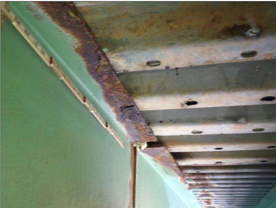
Span 1 Beam 6: 20" OF RUST SCALE ON NORTH AND SOUTH EDGE OF TOP FLANGE WITH 1/8" REMAINING AT BENT 1. (PAR)
