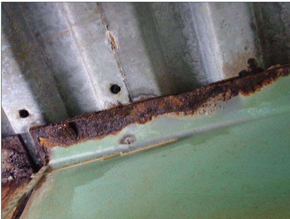
Span 3 Beam 6: 15" x 2 1/2" area of 1/8" section loss (3/8" remaining) on both sides of top flange at Bent 2 (PAR)
