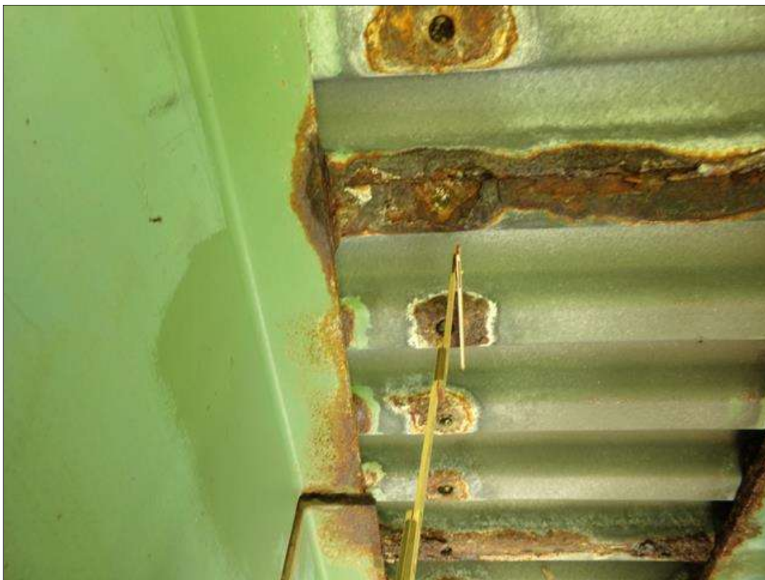
Span 1 Deck: 1/2 SF RUST SCALE WITH 1/8" REMAINING BEAMS 11 AND 12 AT BENT 1. (PAR)
