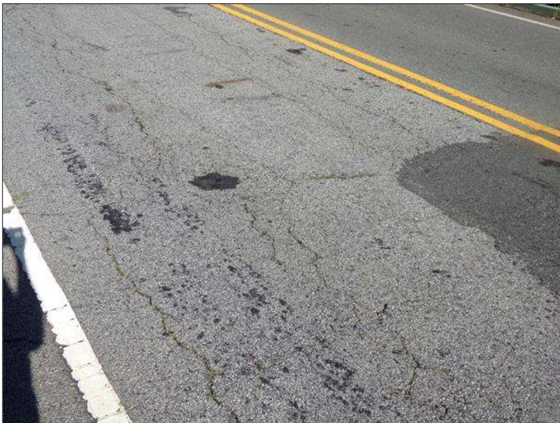
Span 1 Wearing Surface: (2) UP TO 35' x 1/2" LONGITUDINAL CRACKS IN Eastbound LANE.
