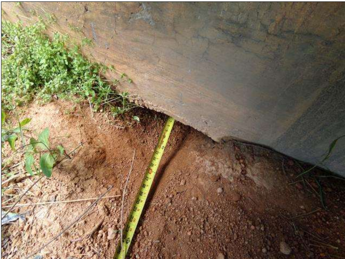
End Bent 1 Abutment: 19" x 12" x 5" high erosion with 9" deep undermining under End Bent 1 cap at East end (PAR)
