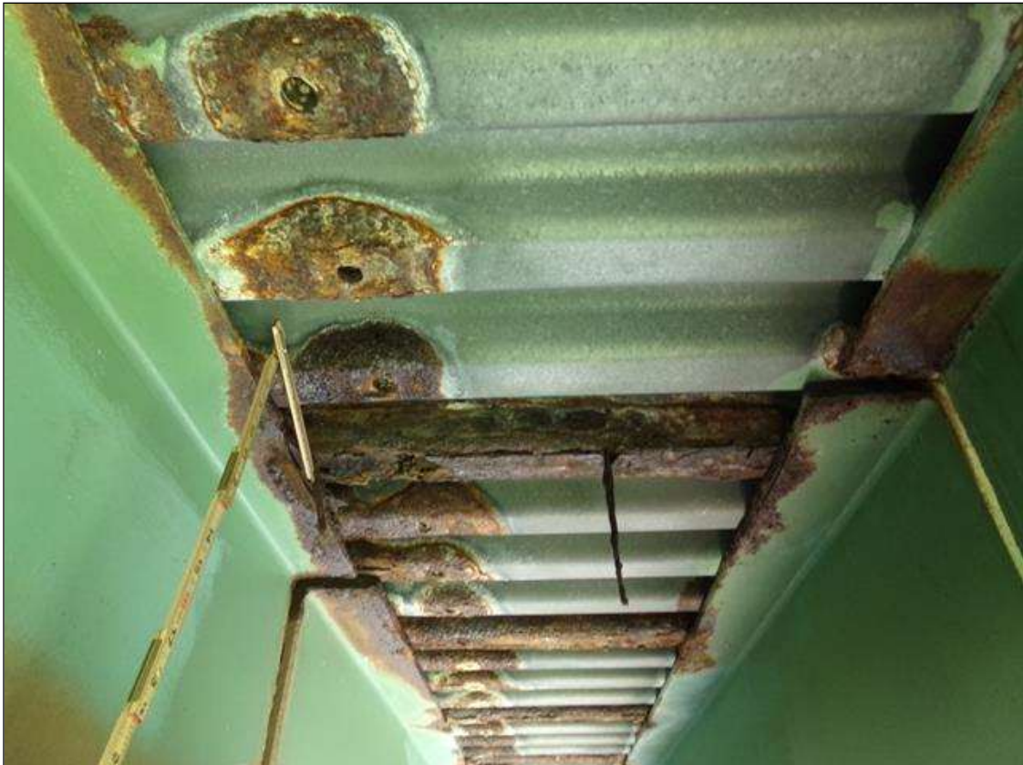
Span 1 Deck: 1 SF RUST SCALE WITH 100% LOSS OF SECTION AND CONCRETE DECK EXPOSED BETWEEN BEAMS 10 AND 11 AT BENT 1. (PAR)
