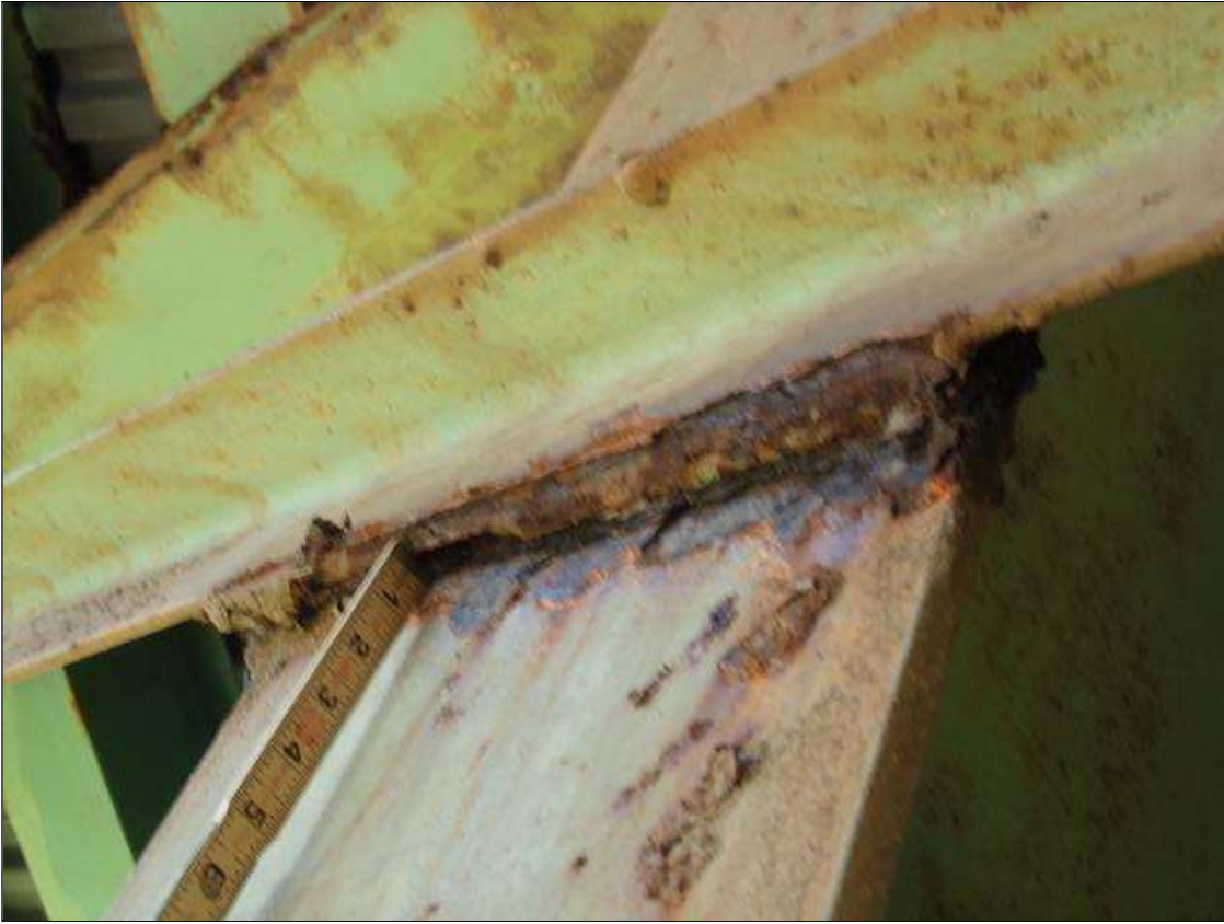
Bent 1 Pile 3: 1" x 10" area of 1/8" section loss (3/8" remaining) on Span 2 flange at diagonal bracing connection (PAR)
