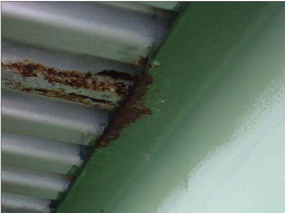
Span 3 Beam 8: 15' OF peeling paint with rust ON TOP AND BOTTOM FLANGES, AT RANDOM THROUGHOUT.
