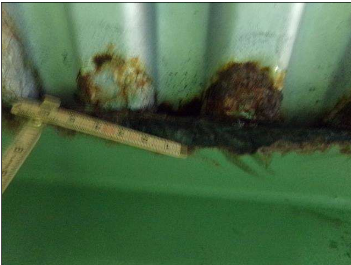
Span 3 Beam 12: 6" x 2" area of 1/8" section loss (3/8" remaining) on both sides of top flange, 9' from End Bent 2 (PAR)
