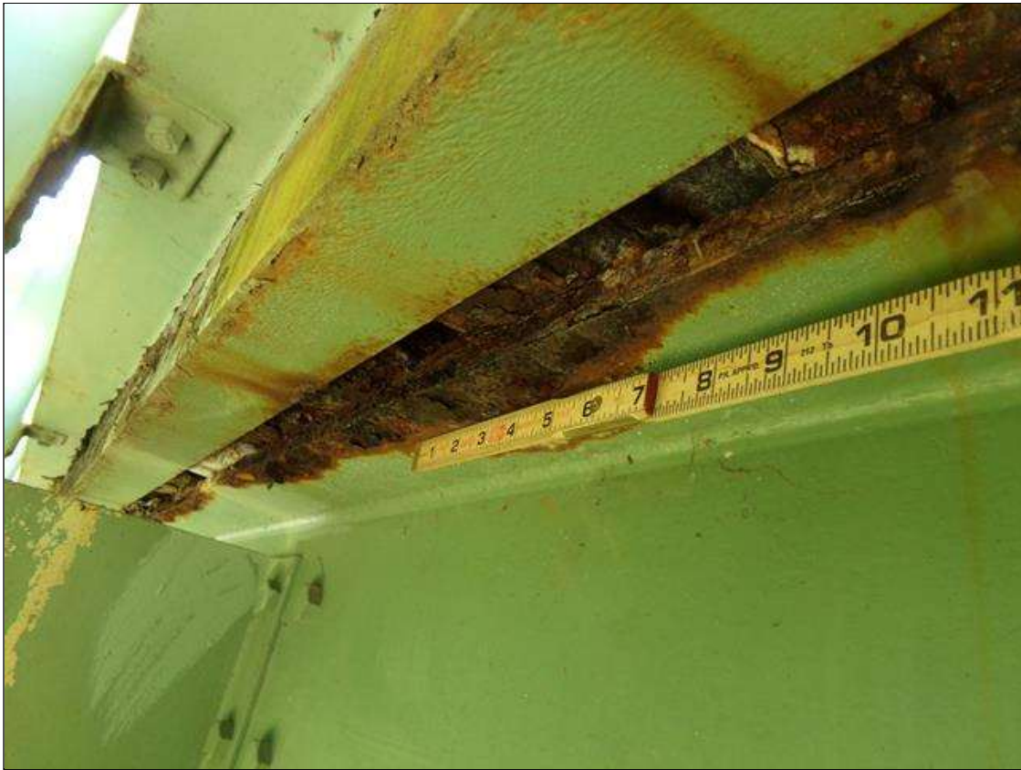
Span 1 Beam 1: 7' x 1" area of 1/16" section loss (7/16" remaining) on left side of top flange near midspan
