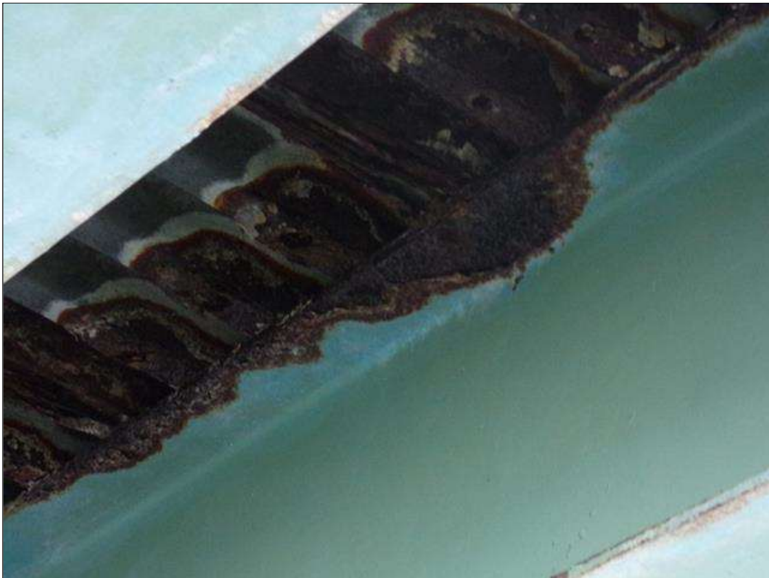
Span 3 Beam 6: 32" x 3" area of 1/8" section loss (3/8" remaining) on right side of top flange, 10' from Bent 2 (PAR)
