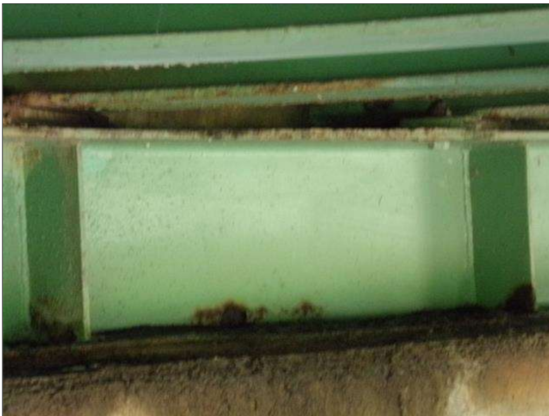
End Bent 2 Cap 1: 15' surface rust on both flanges
