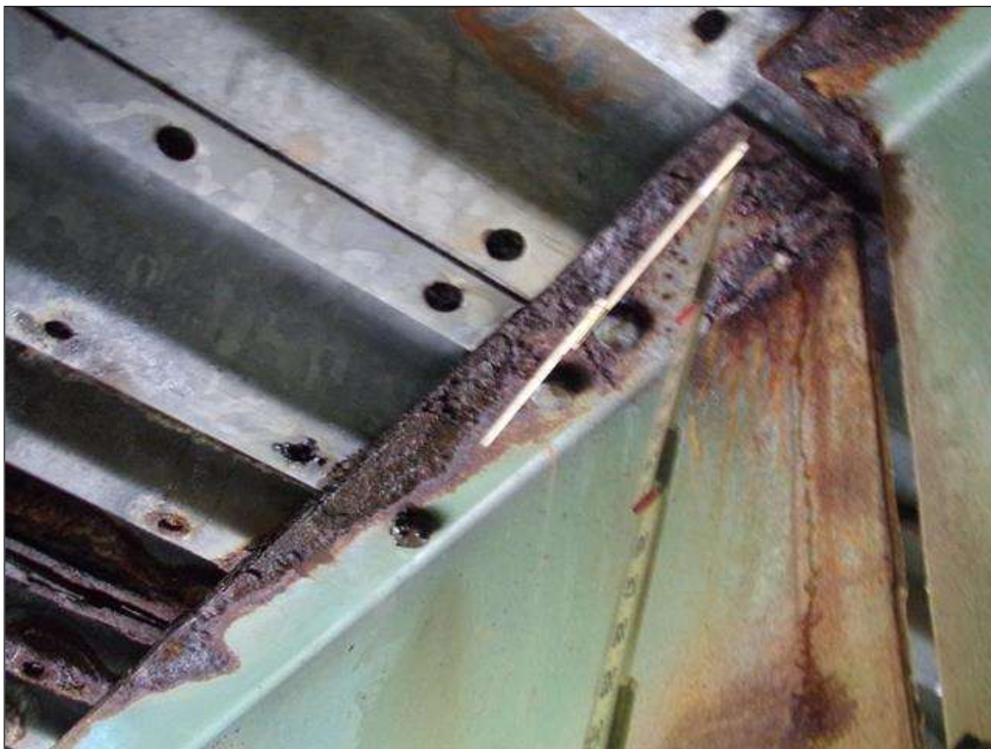
Span 2 Beam 6: 30" x 3" area of 1/8" section loss (3/8" remaining) on right side of top flange at Bent 2 (PAR)
