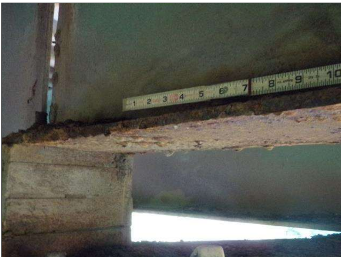
Span 1 Beam 7: 18" x 3" area of 1/8" section loss (3/8" remaining) on both sides of bottom flange at Bent 1 (PAR)
