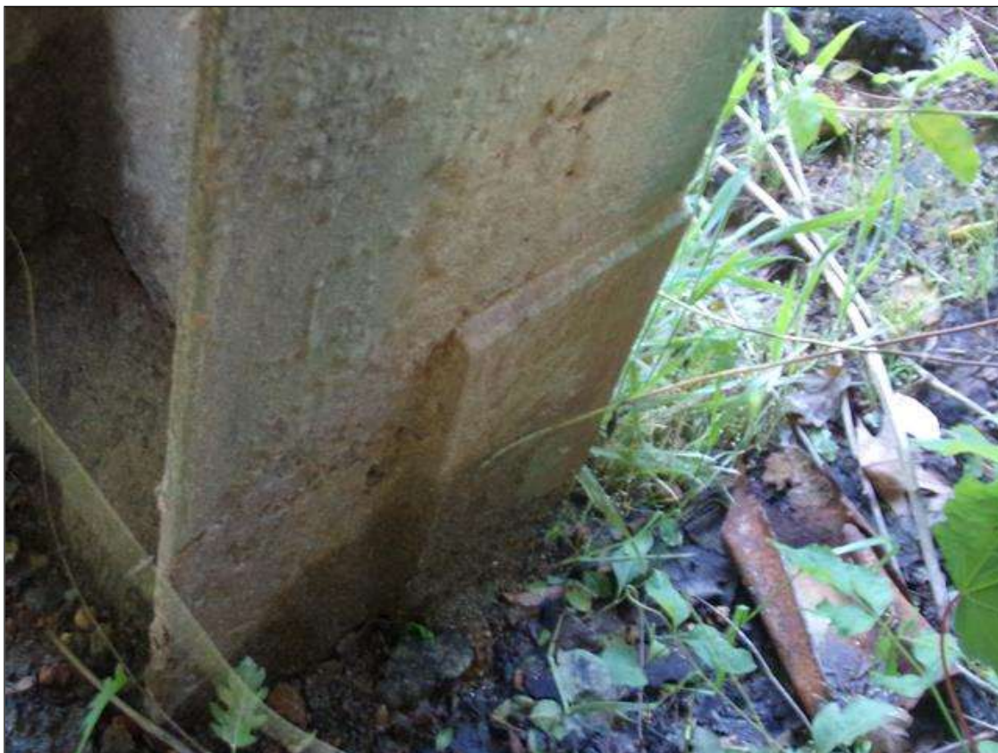
BENT 1 PILE 3: 1' x 6" x 1/4" WELDED REPAIR PLATE ON THE WEST FACE AT BOTTOM OF PILE.
