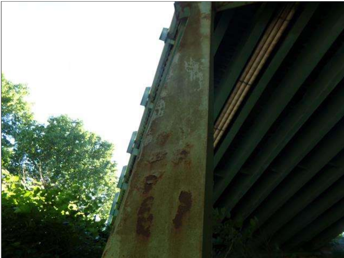
Bent 2 Pile 1: 8' OF FRECKLED RUST WITH ISOLATED LOCATIONS SURFACE RUST ON ALL SURFACES, AT RANDOM THROUGHOUT.
