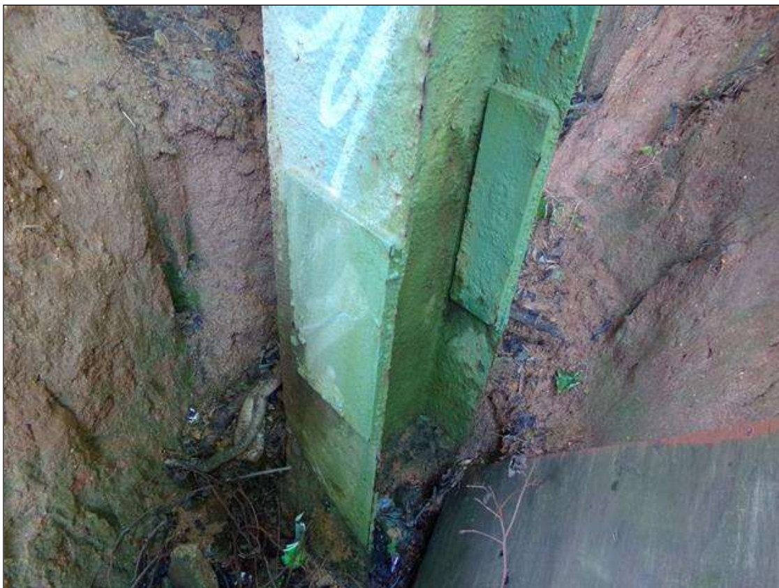
BENT 1 PILE 1: (3) UP TO 16" x 9" x 1/4" WELDED REPAIR PLATES ON EAST AND WEST FLANGES, 14' FROM BOTTOM OF CAP. (PHOTO TAKEN ON EAST FLANGE)
