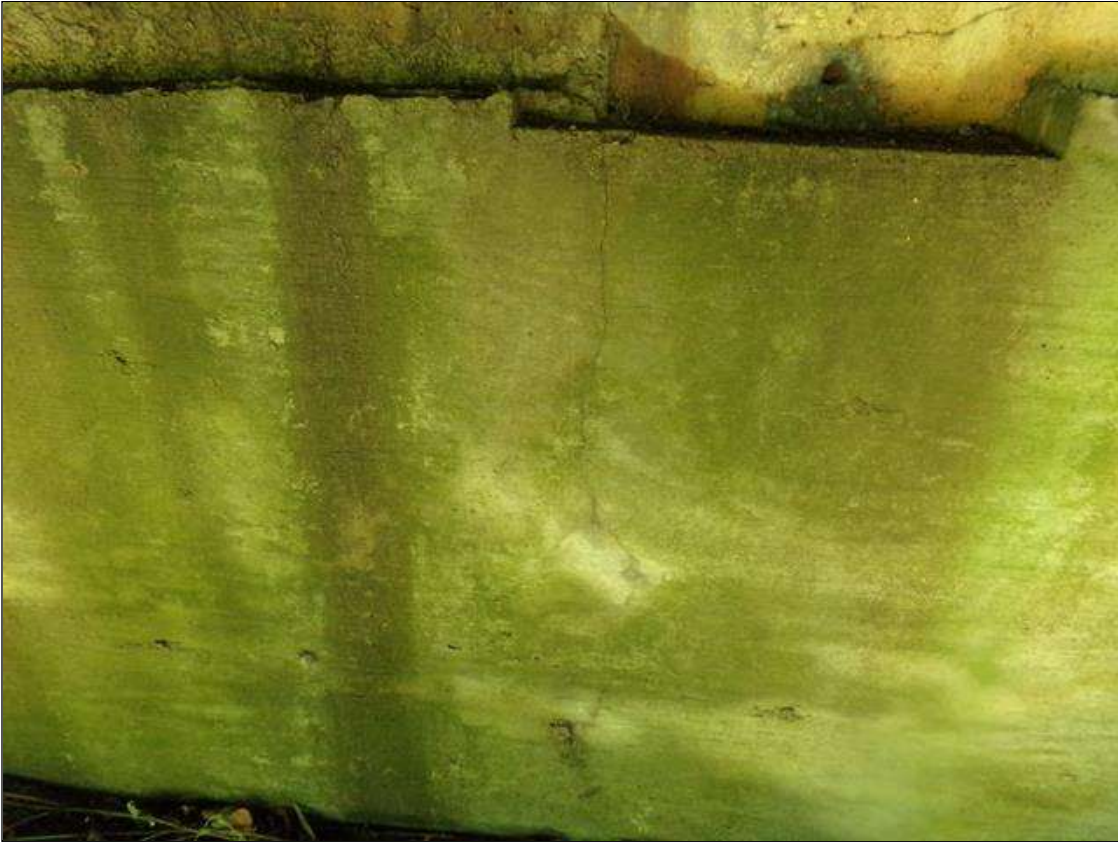
End Bent 2 Abutment: (4) UP TO 2 1/2' x 1/32" VERTICAL CRACKS AT RANDOM THROUGHOUT WEST FACE OF ABUTMENT. (PHOTO TAKEN BENEATH BEAM 10)
