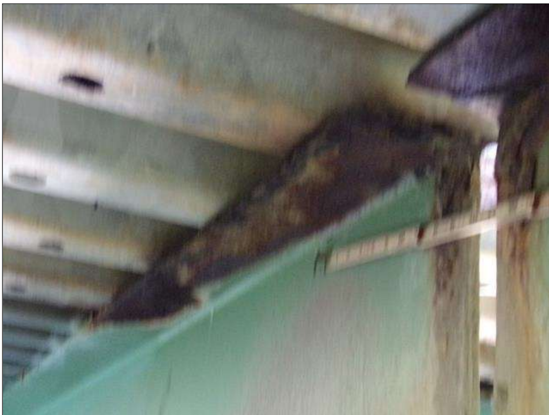
Span 2 Beam 7: 24" x 4" area of 1/4" section loss (1/4" remaining) on both sides of top flange at Bent 1 (PAR)
