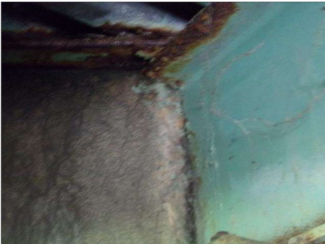
End Bent 1 Abutment: (12) UP TO 18" x UP TO 3" x 1" SPALLS ON SOUTH BEAM INTERFACE IN ABUTMENT BACKWALL AT ALL BEAM ENDS. (PHOTO TAKEN IN BETWEEN BEAMS 5 AND 6)
