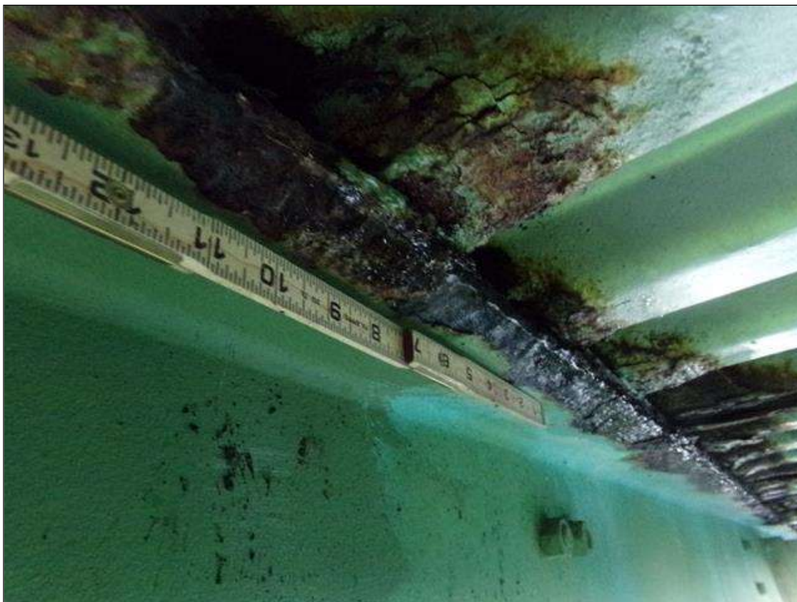
Span 3 Beam 12: 20" x 1 1/2" area of 1/8" section loss (3/8" remaining) on both sides of top flange, 11' from End Bent 2 (PAR)
