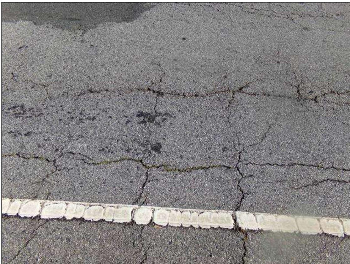
Span 1 Wearing Surface: 45 square feet up to 1/4" transverse cracks
