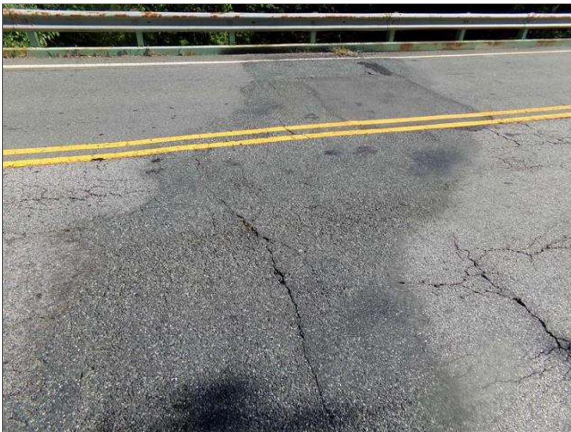
Span 2 Wearing Surface: 27' x UP TO 5' PATCHED AREA AT BENT 2 JOINT.
