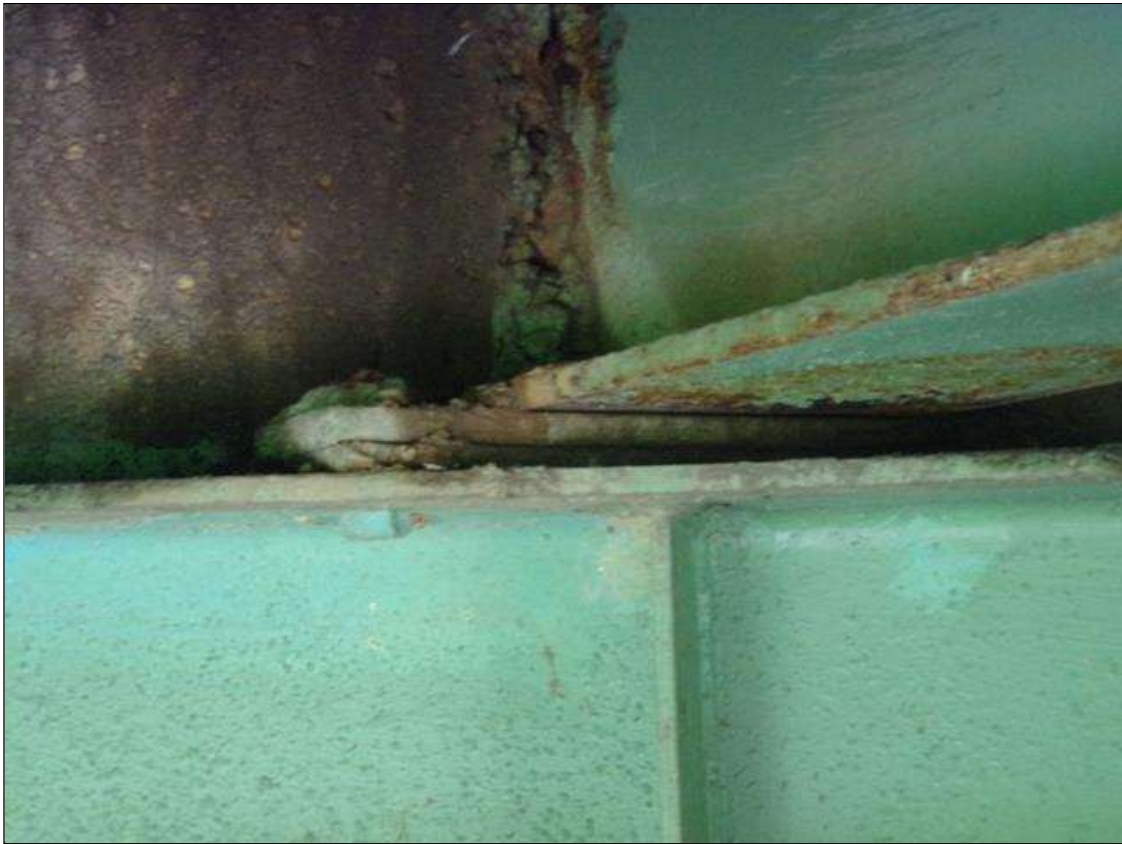
Span 3 Far Bearing: surface rust
