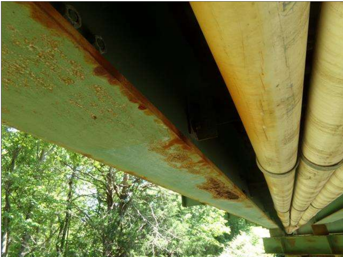
Span 1 Beam 1: 20' OF LIGHT SCALING WITH ISOLATED LOCATIONS SURFACE RUST ON TOP AND BOTTOM FLANGES, AT RANDOM THROUGHOUT. (PHOTO TAKEN NEAR MID Span)
