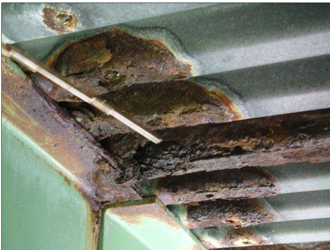
Span 1 Deck: 1 SF RUST SCALE WITH 100% LOSS OF SECTION AND CONCRETE DECK EXPOSED BETWEEN BEAMS 9 AND 10 AT BENT 1. (PAR)
