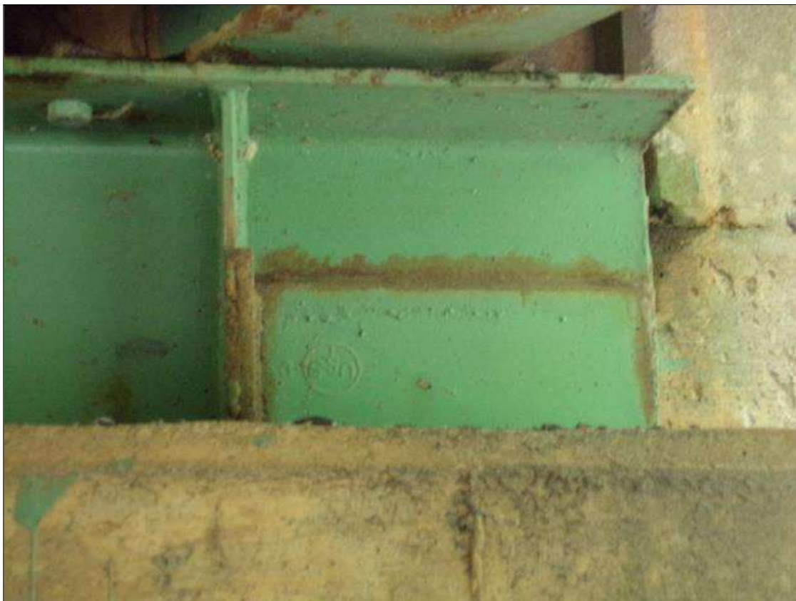
End Bent 1 CAP: 13" x 5" x 6" x 1/2" ANGLE REPAIR AT NORTH END.
