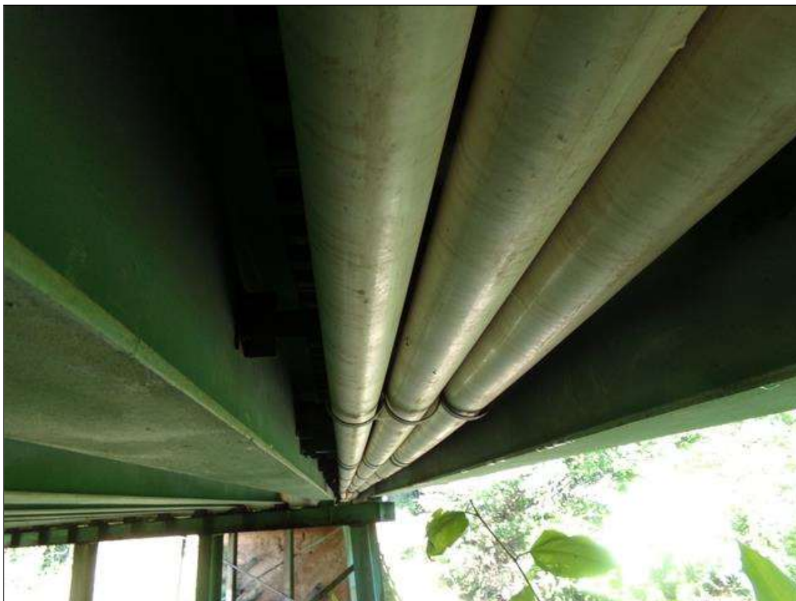
(3) 4" diameter utilities in Bay 1
