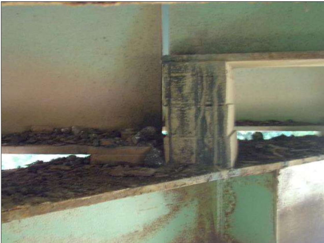
Bent bearing (Beam 8, Bent 1 shown)
