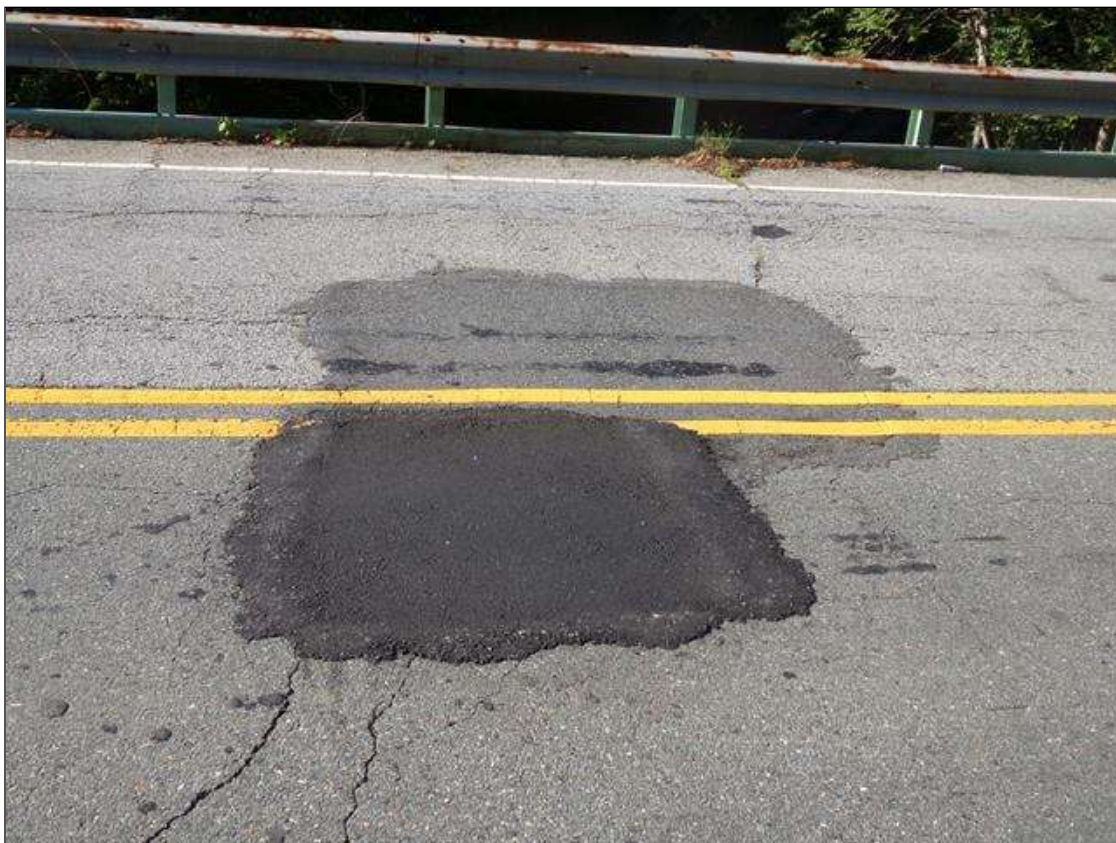
Span 2 Wearing Surface: 7' x 5' PATCHED AREA AT CENTERLINE OF ROADWAY AT BENT 1.
