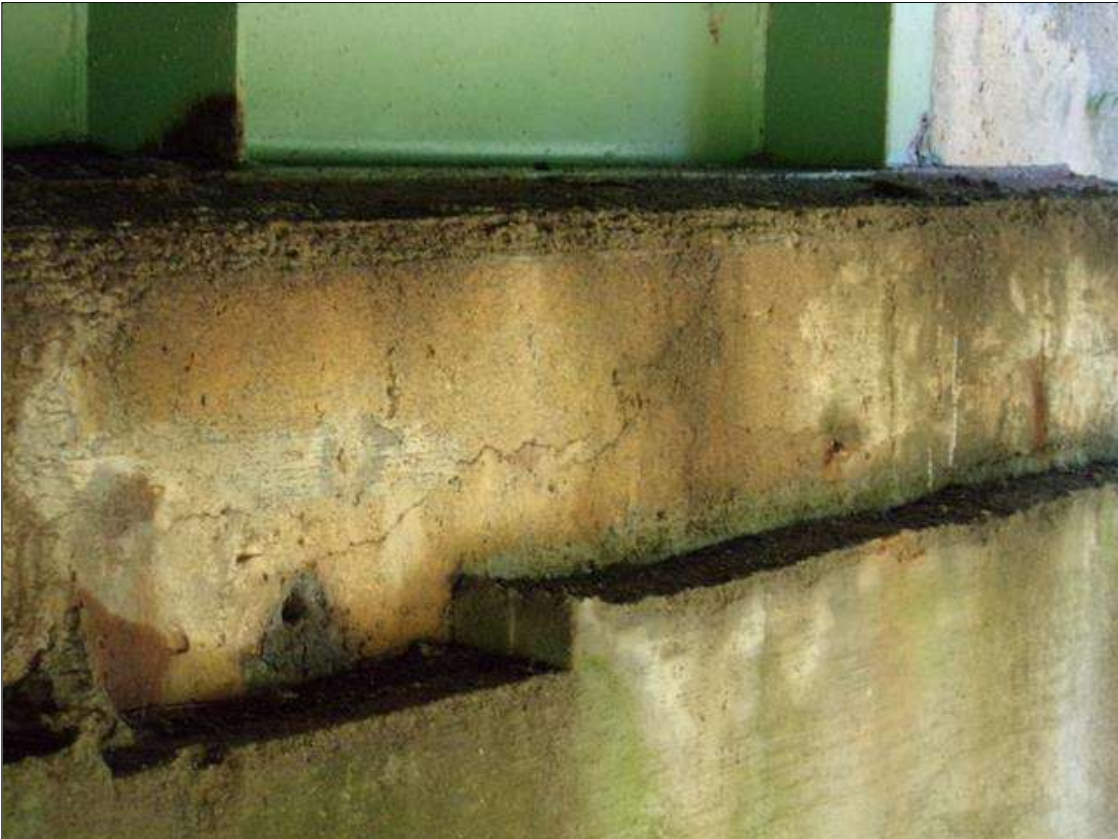
End Bent 2 Abutment: 15' x UP TO 1/32" HORIZONTAL ON WEST FACE OF UPPER ABUTMENT WALL BETWEEN BEAMS 8 THROUGH 11.
