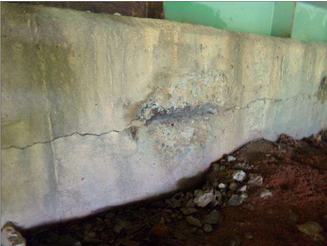
End Bent 1 Abutment: 16" x 9" x UP TO 1 1/2" SPALL, WITH EXPOSED REINFORCING, WITH 20% LOSS OF SECTION OF EXPOSED REINFORCING.
