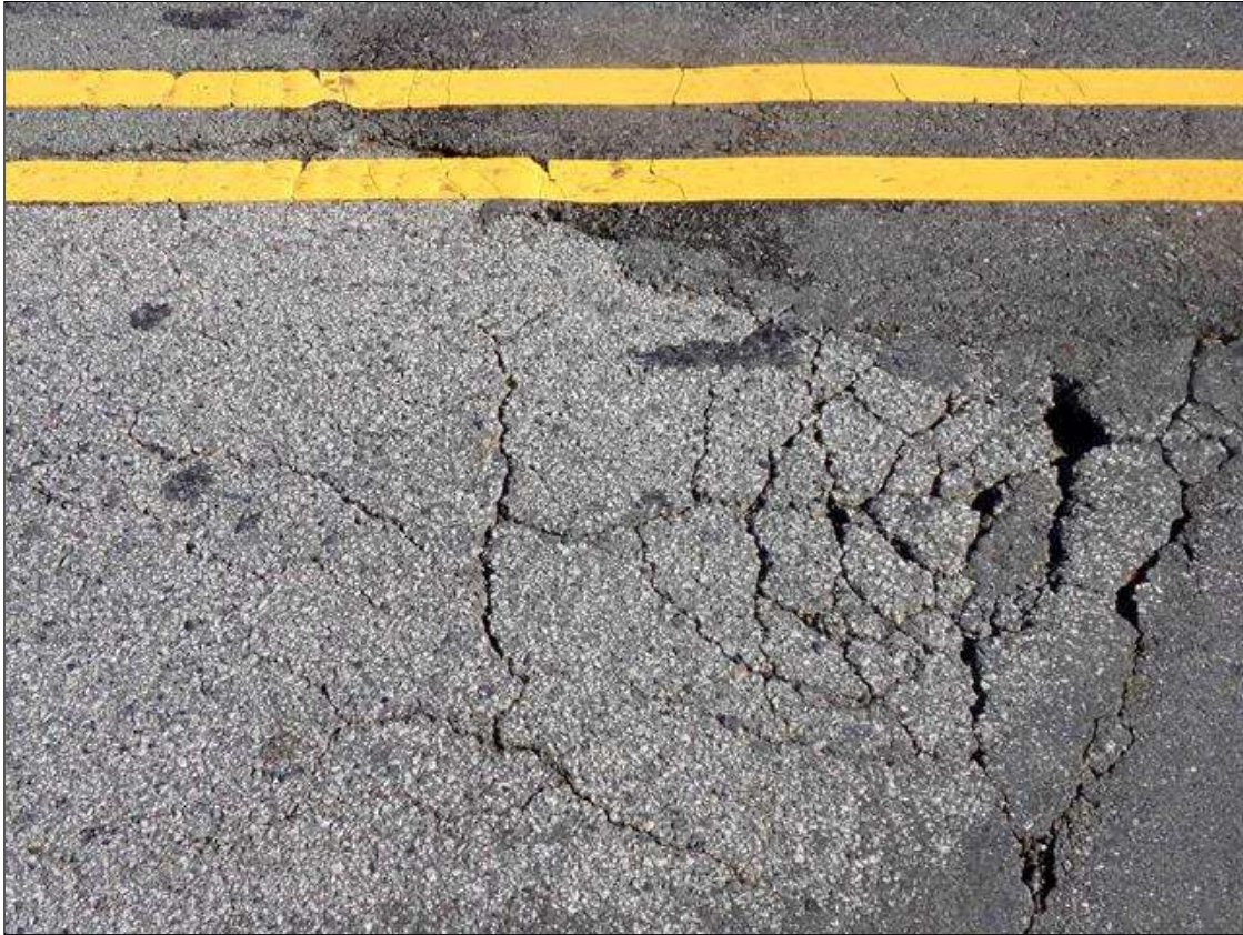
Span 3 Wearing Surface: MAP CRACKING UP TO 1/4" AT RANDOM THROUGHOUT ASPHALT WEARING SURFACE. (PHOTO TAKEN IN Eastbound LANE 1' FROM END BENT 2)
