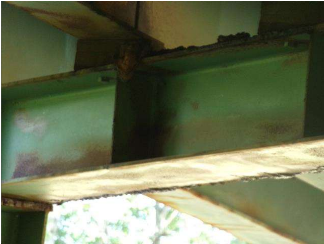
Bent 2 Cap 1: 25' OF SURFACE RUST WITH ISOLATED LOCATIONS FRECKLED RUST ON TOP AND BOTTOM FLANGES AND UP TO 5" IN WEB, AT RANDOM THROUGHOUT EAST AND WEST FACES.
