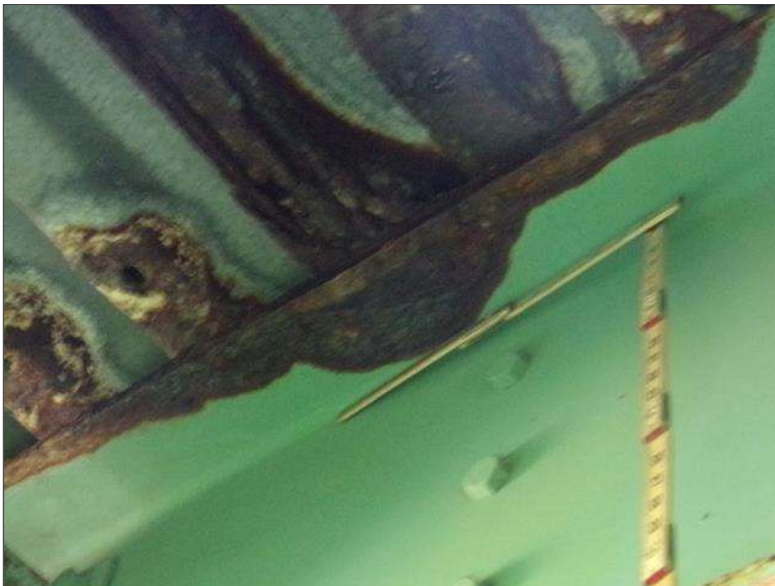
Span 3 Beam 11: 7' x 2" area of 1/8" section loss (3/8" remaining) on both sides of top flange near midspan (PAR)
