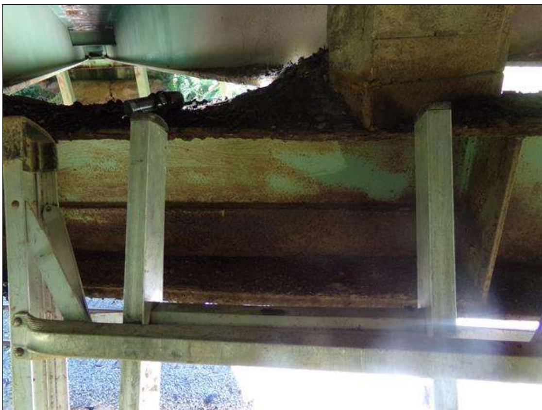
BENT 1 CAP: 29" x 5" x 4.5" x 1/2" THICK CAP REPAIR BETWEEN BEAMS 6 AND 7.
