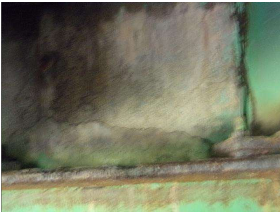
End Bent 1 Abutment: 8' x UP TO 1/16" HORIZONTAL CRACK IN ABUTMENT BACKWALL BETWEEN BEAMS 5 AND 7. (PHOTO TAKEN IN BETWEEN BEAMS 5 AND 6)
