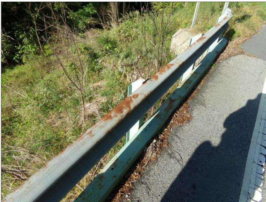
Span 1 Right Bridge Rail: SURFACE RUST AT RANDOM THROUGHOUT GUARDRAIL AND CURB RAIL.
