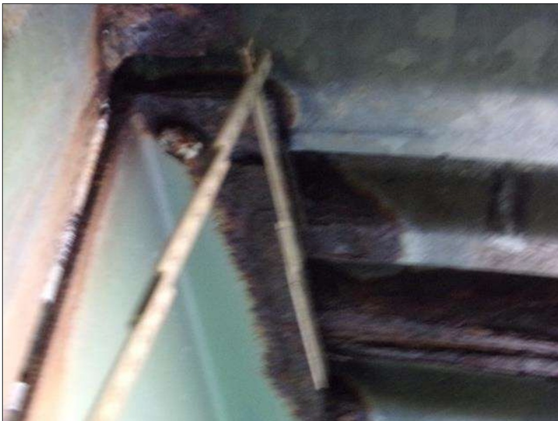
Span 2 Beam 7: 20" x 2" area of 1/8" section loss (3/8" remaining) on both sides of top flange at Bent 2 (PAR)
