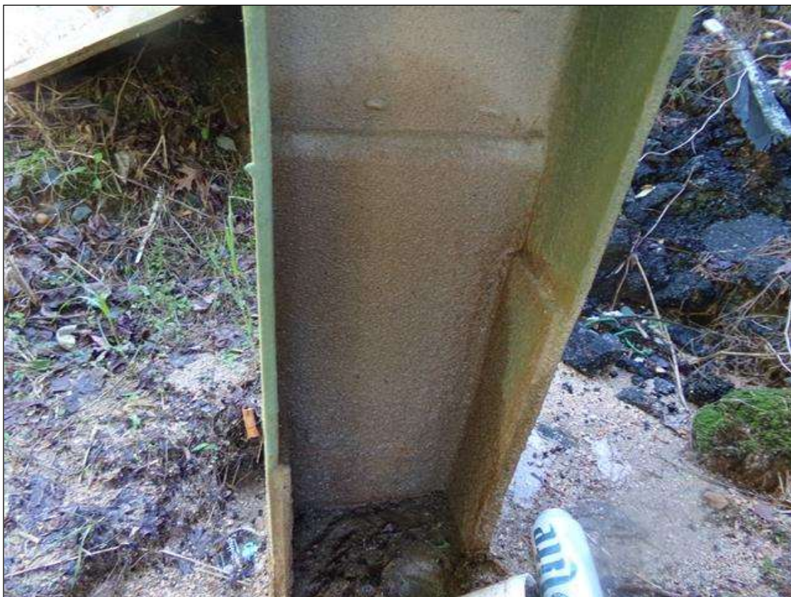
BENT 2 PILE 1: (4) UP TO 2' x 10" x 1/2" WELDED REPAIR PLATES ON NORTH AND SOUTH FACES, AT SOIL INTERFACE. (PHOTO TAKEN NORTH FACE)
