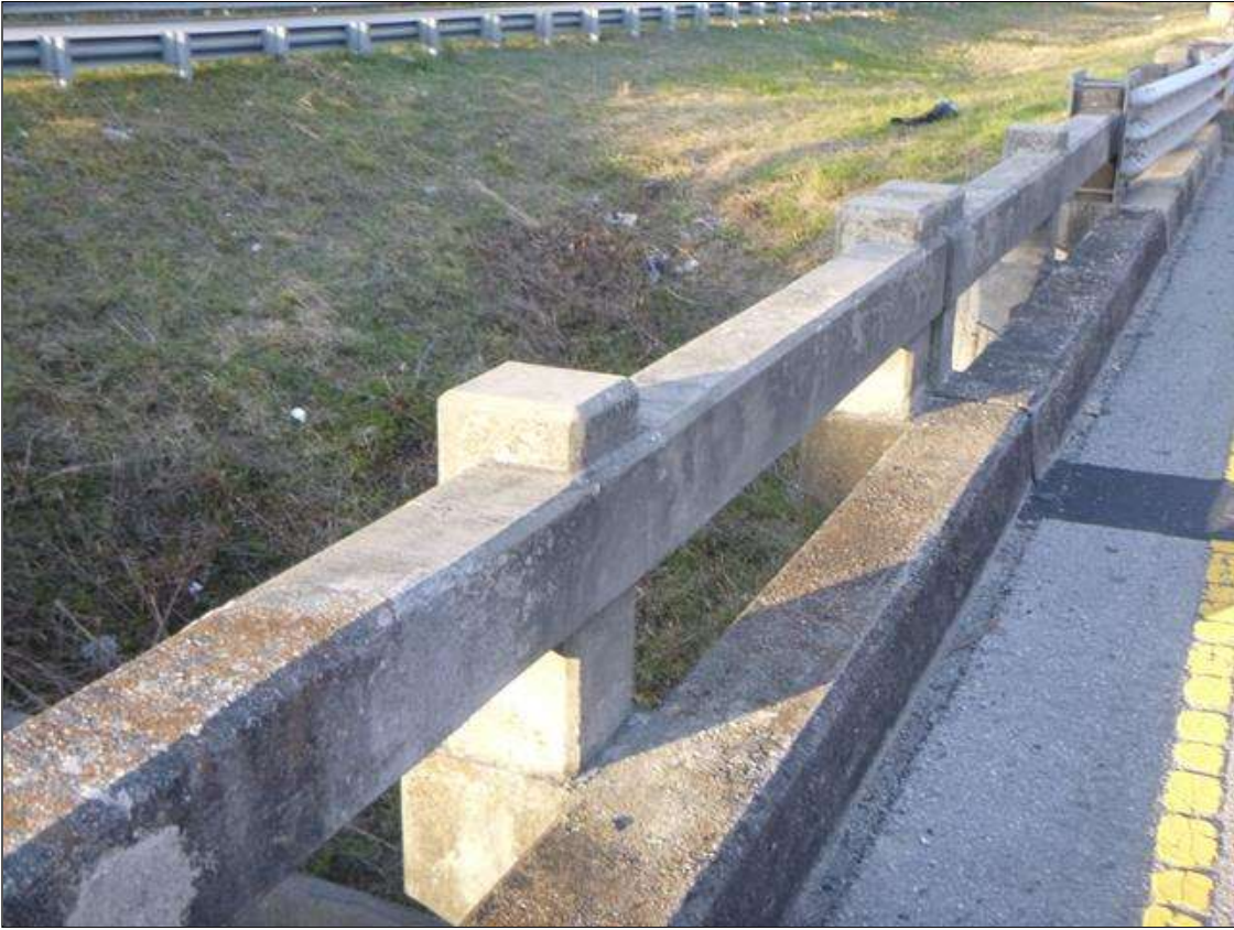
Span 2 Left Bridge Rail: PATCHED AREA IN LEFT RAIL, SPAN 2 (14' LONG)
