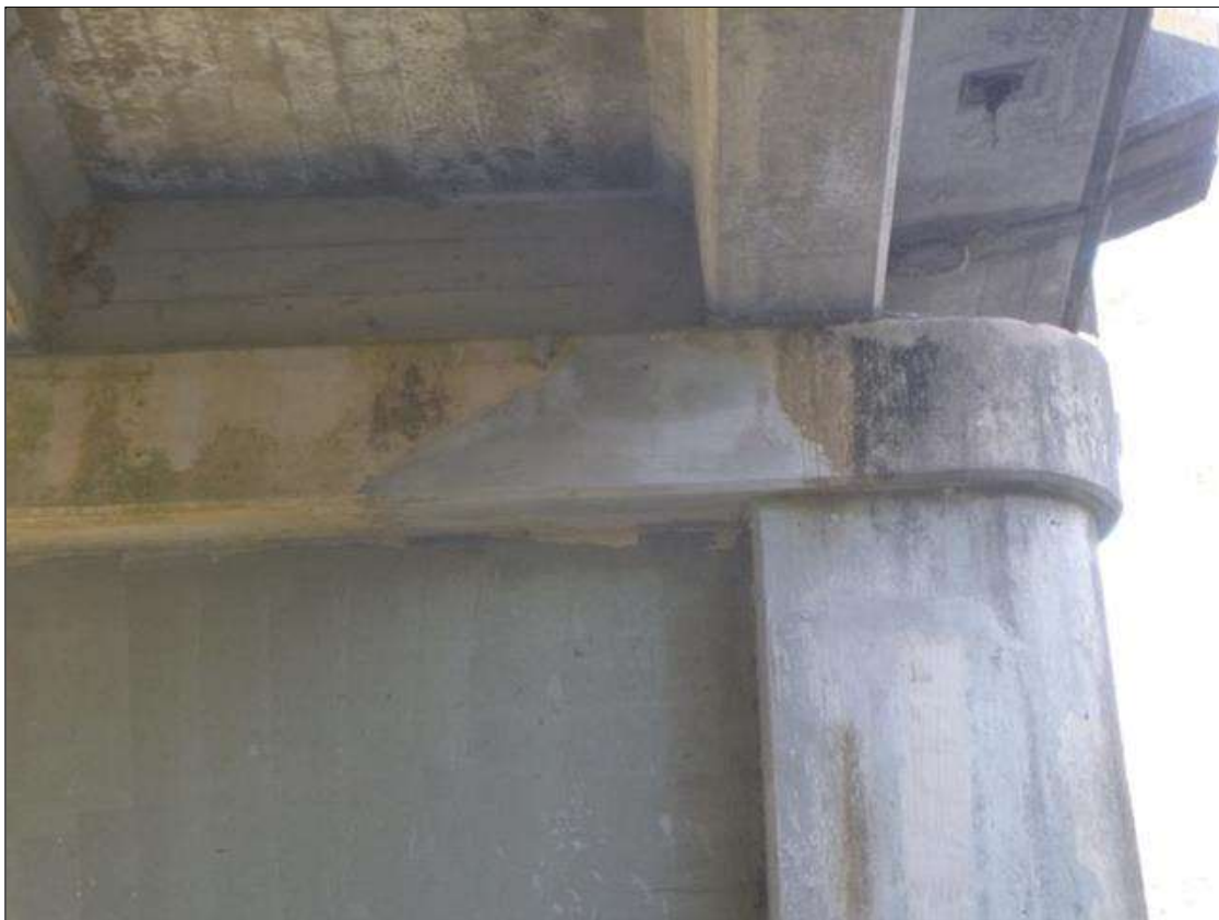
Bent 2 Cap 1: SOUND PATCHED AREA IN PIER 2 CAP SPAN 2 SIDE UNDER BAY 3, 3' LONG X 18" HIGH)
