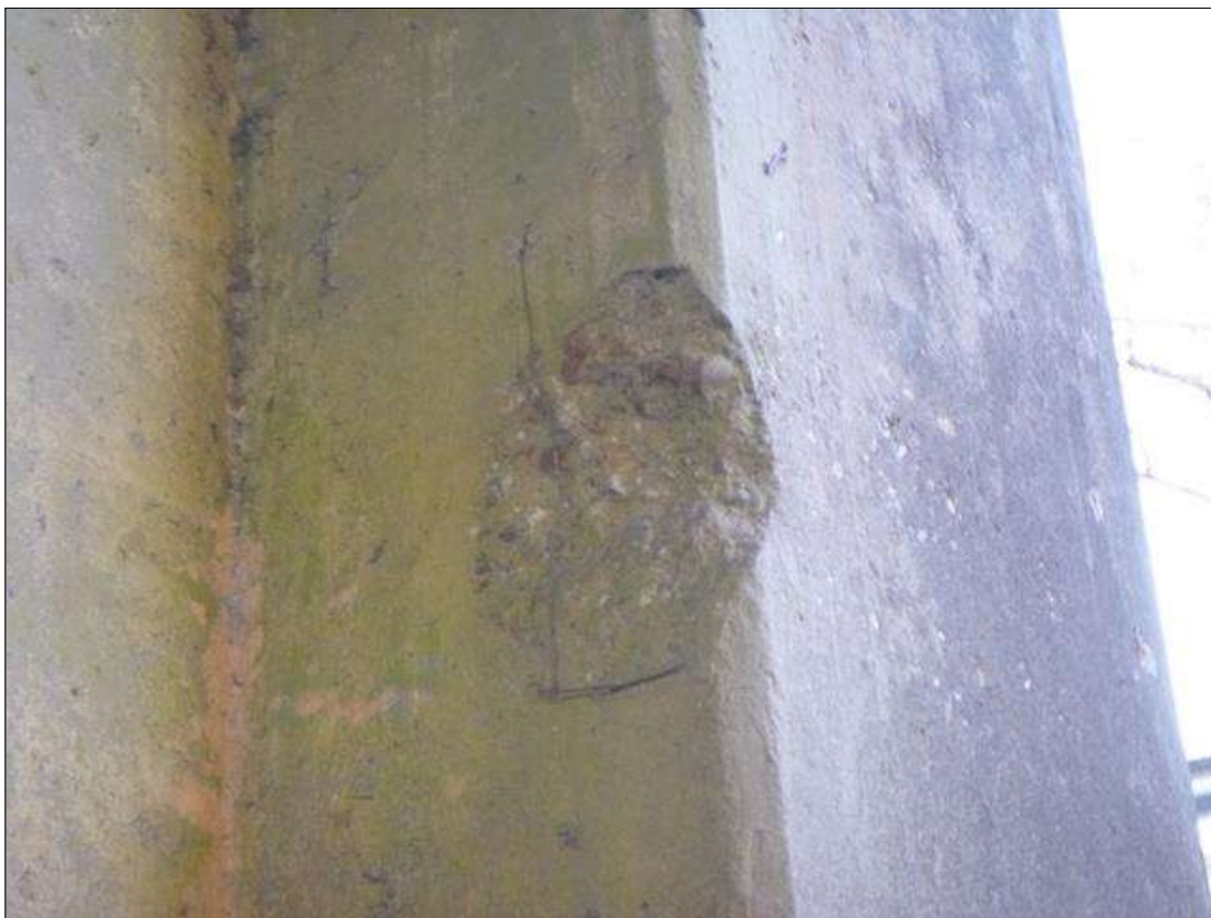
Bent 1 Pier 1: 9" DIAMETER X 1" DEEP SPALL IN NOSE PORTION NORTH FACE AT WEST END
