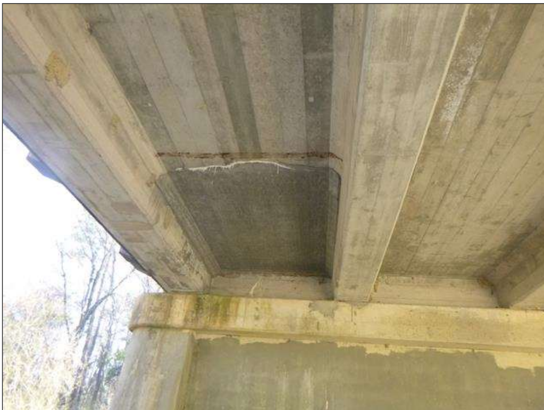
Span 3 Deck: SPAN 3 DECK UNDERSIDE IN BAY 3 PATCHED AREA AT PIER 2, 10' LONG X 5' WIDE.
