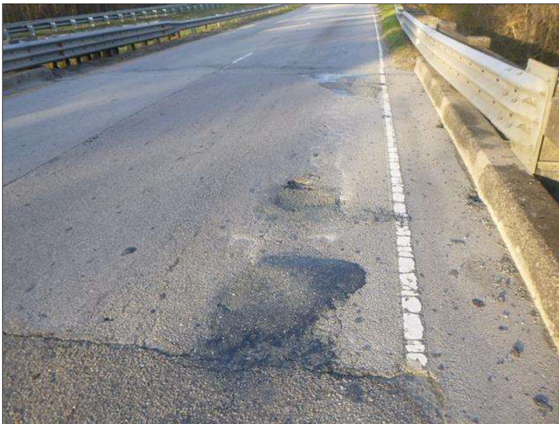
Span 3 Wearing Surface: 4 SOUND PATCHED AREAS IN RIGHT TRAVEL LANE UP TO 2.5' X 1.5'
