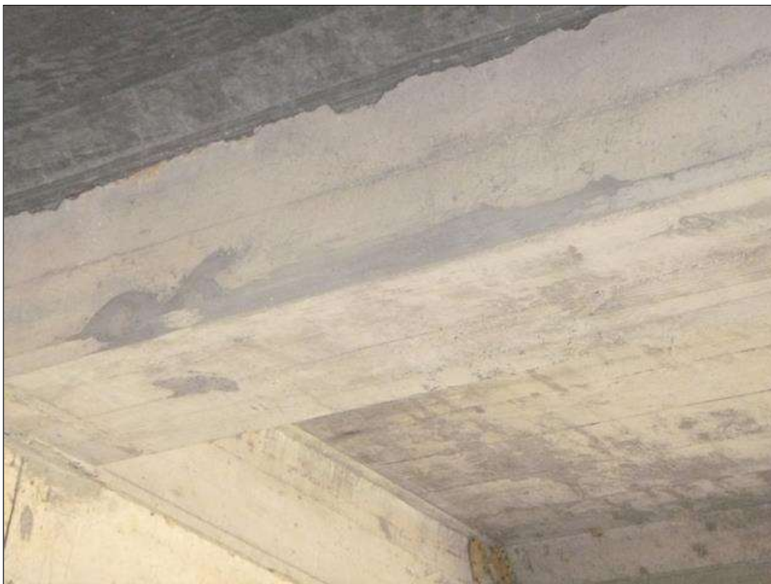
Span 3 Beam 3: GIRDER 3 IN SPAN 3 AT PIER 2 BAY 3 SIDE LONGITUDINAL CRACKING 3' LONG THAT HAS BEEN PATCHED AND IS SOUND
