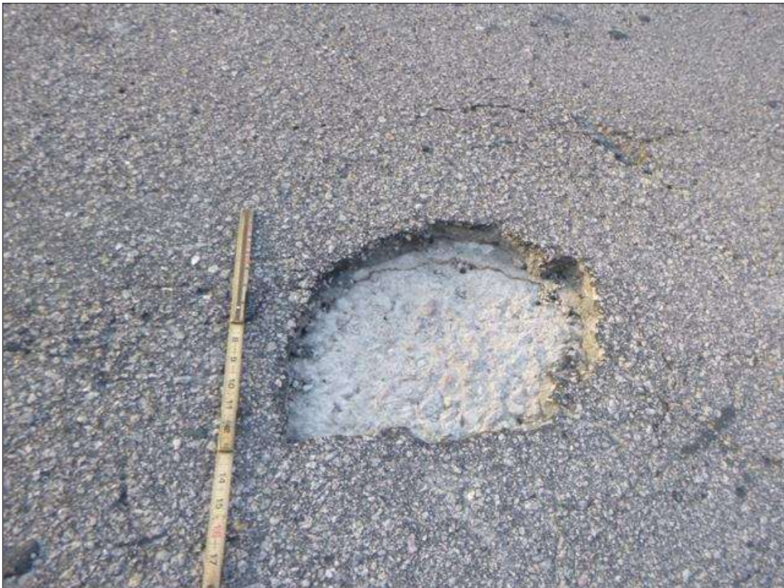
Span 1 Wearing Surface: (PAR) 17" X UP TO 12" X FULL DEPTH POT HOLE, 3' FROM ABUTMENT 1 AND 5' FROM EAST BRIDGE RAIL.
