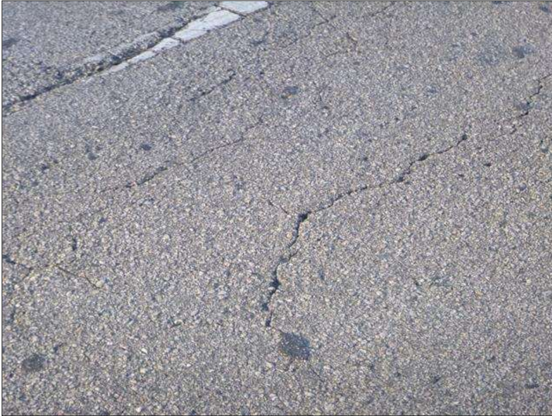
Span 1 Wearing Surface: SCATTERED HAIRLINE TO 1/8" WIDE MAP CRACKING IN ASPHALT WEARING SURFACE
