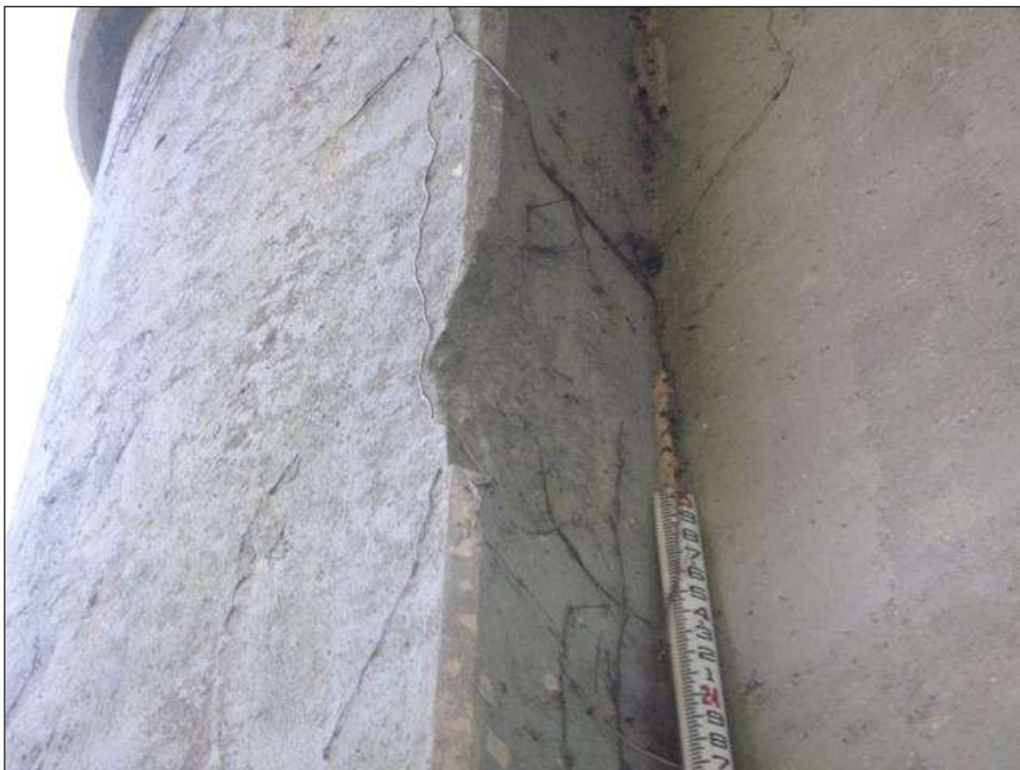
Bent 1 Pier 1: 16" X 9" X 1" DEEP SPALL IN NOSE PORTION NORTH FACE AT EAST END
