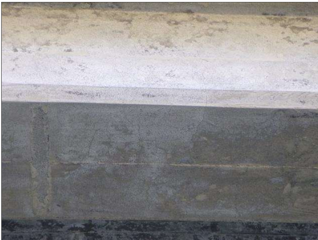
Span 1 Beam 4: 5' OF HAIRLINE TRANSVERSE / MAP CRACKING RIGHT OF MID SPAN TOWARDS PIER 1
