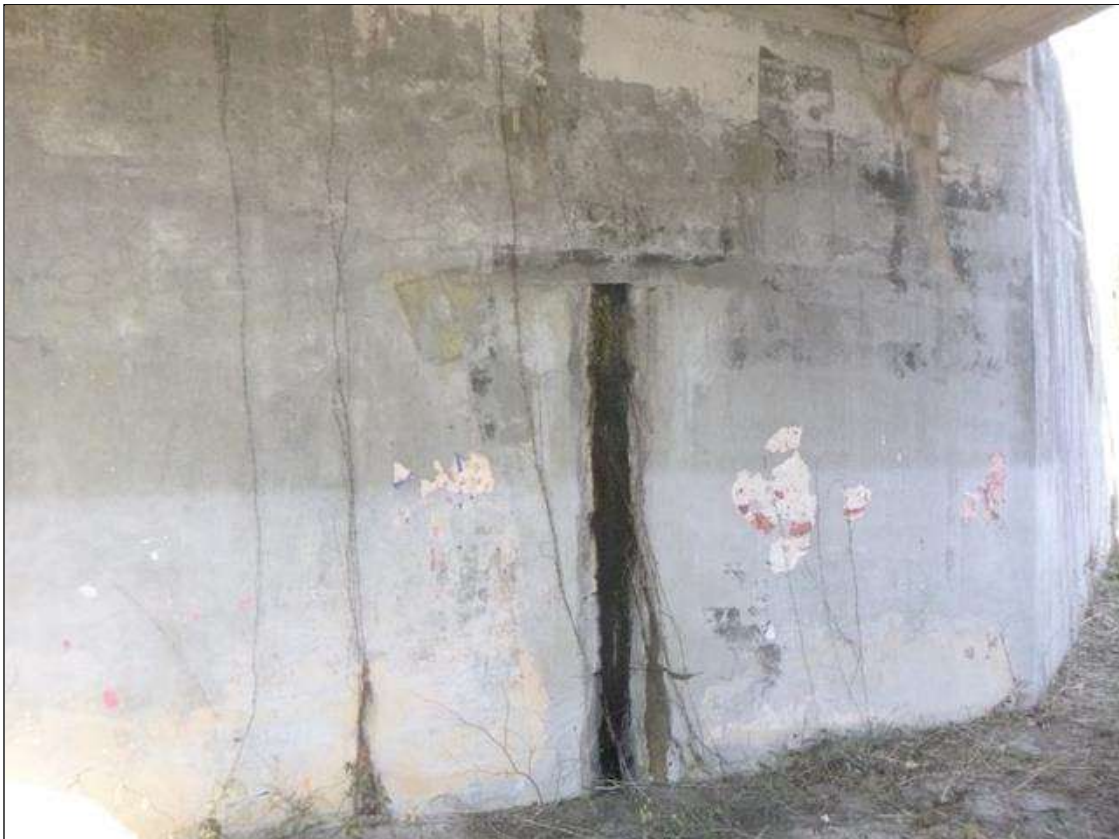
Abutment 2 Abutment: DIAGONAL / HORIZONTAL / VERTICAL CRACKING UP TO 1/32" WIDE ALONG THE ABUTMENT 2 BREASTWALL AT LOWER PORTION WITH RUST LEAKAGE.
