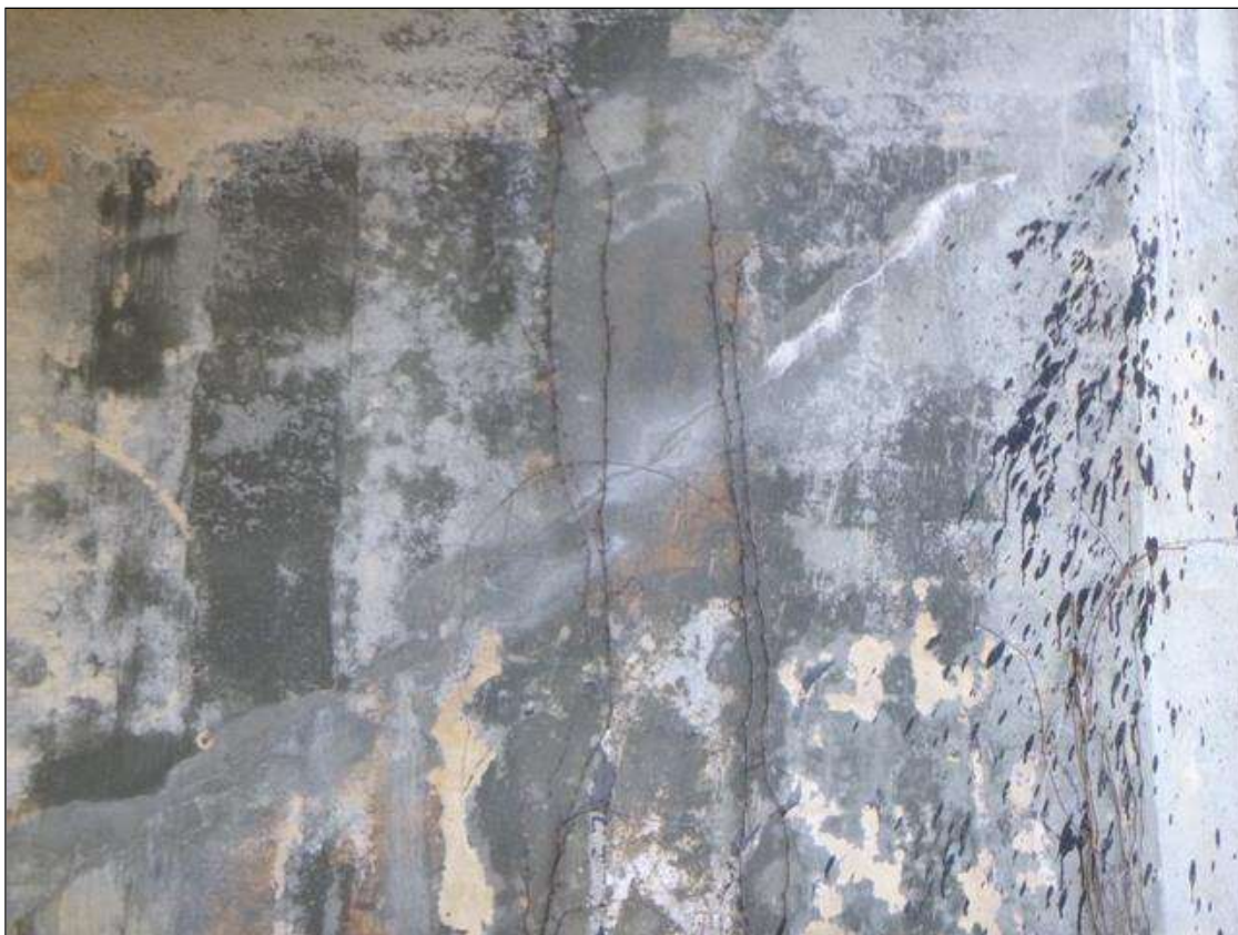
Abutment 1 Abutment: HORIZONTAL/DIAGONAL CRACKING WITH EFFLORESCENCE ALONG THE ABUTMENT 1 BREASTWALL (25' LONG X UP TO 1/8" WIDE)
