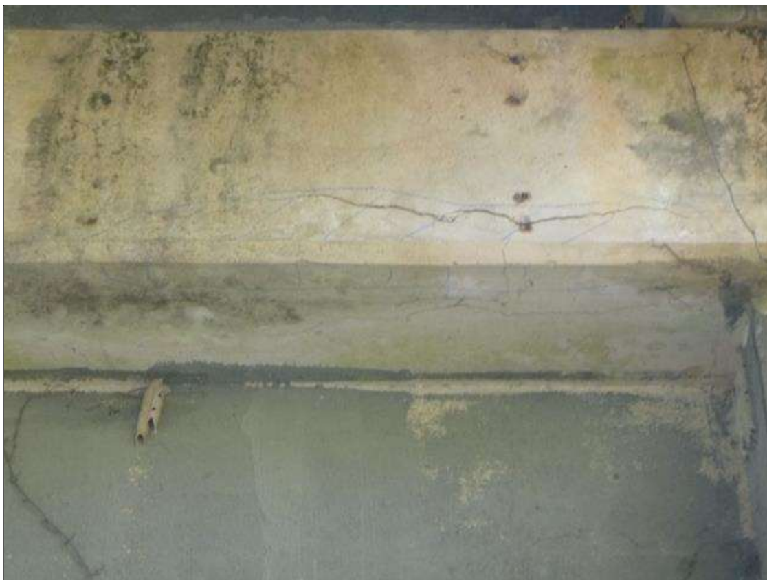
Bent 1 Cap 1: UP TO 1/8" HORIZONTAL CRACK AND DELAMINATED AREA IN PIER 1 CAP SOUTH SIDE UNDER BAY 3 (2' LONG X 4" HIGH)
