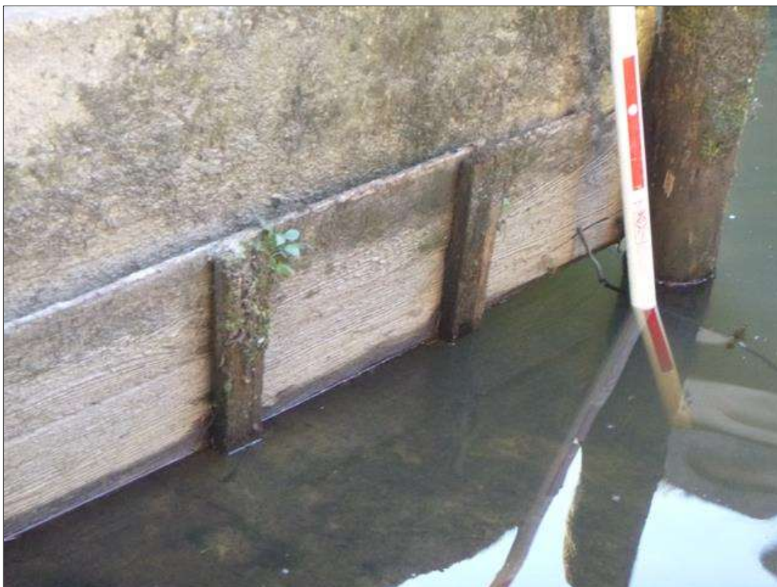
Bent 2 Footing: (PAR) SCOUR AROUND FOOTING FULL LENGTH EXPOSING FOOTING WITH 1' OF UNDERMINING FULL WIDTH AT UPSTREAM END
