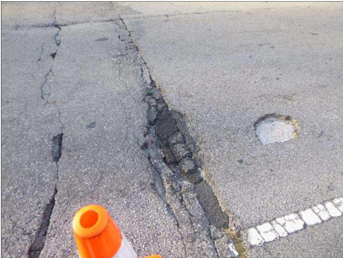
Span 1 Wearing Surface: UP TO 1/2" TRANSVERSE CRACKING AND 4' X UP TO 1' X 2" CRACKED PATCHED AREA IN EAST LANE IN ASPHALT WEARING SURFACE OVER ABUTMENT 1.
