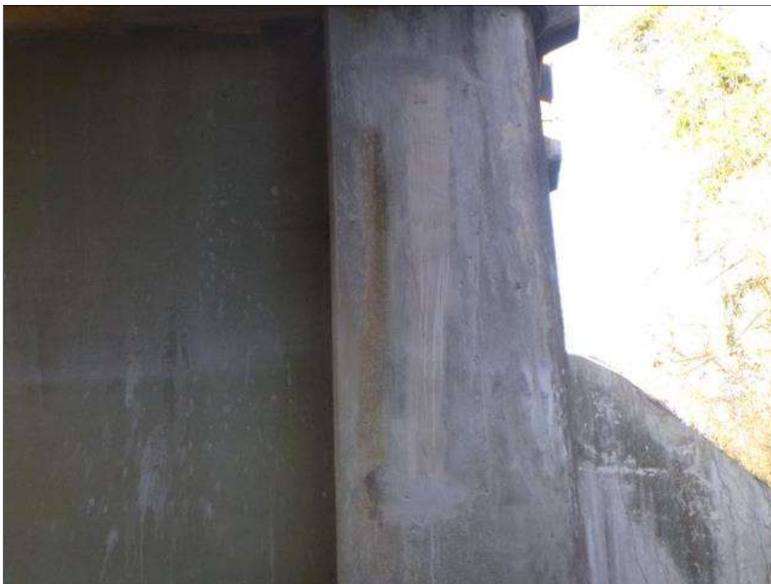
Bent 2 Pier 2: SOUND PATCHED AREA ON NOSE PORTION PIER 2 SPAN 2 SIDE 7" WIDE X 8' HIGH UNDER BEAM 4.
