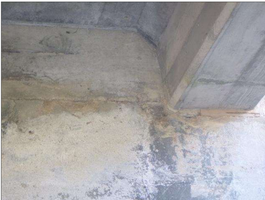
Abutment 1 Abutment: 2 SMALL SPALLS UP TO 6" X 4" X 1" DEEP AT TOP UNDER BAY 1
