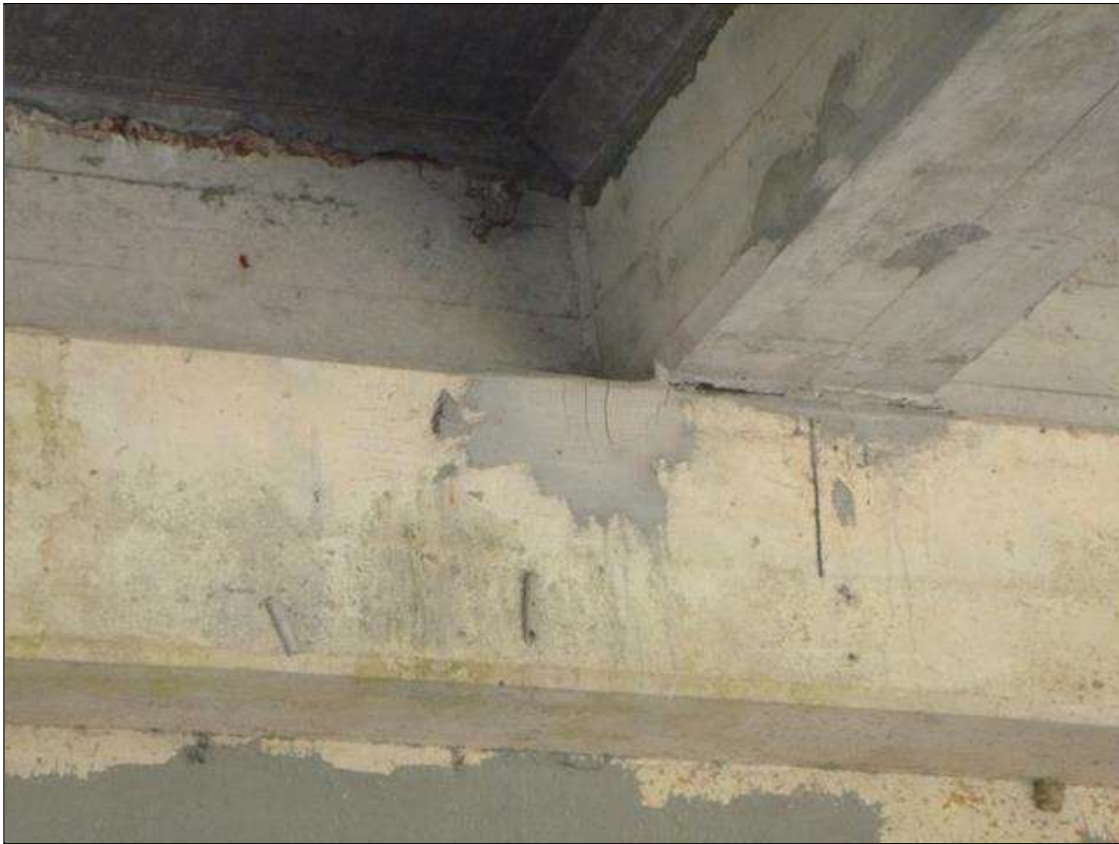
Bent 2 Cap 1: CRACKED PATCHED AREA WITH UP TO 1/16" CRACKING IN PIER 2 CAP SPAN 3 SIDE UNDER BAY 3, 9" LONG X 9" HIGH)
