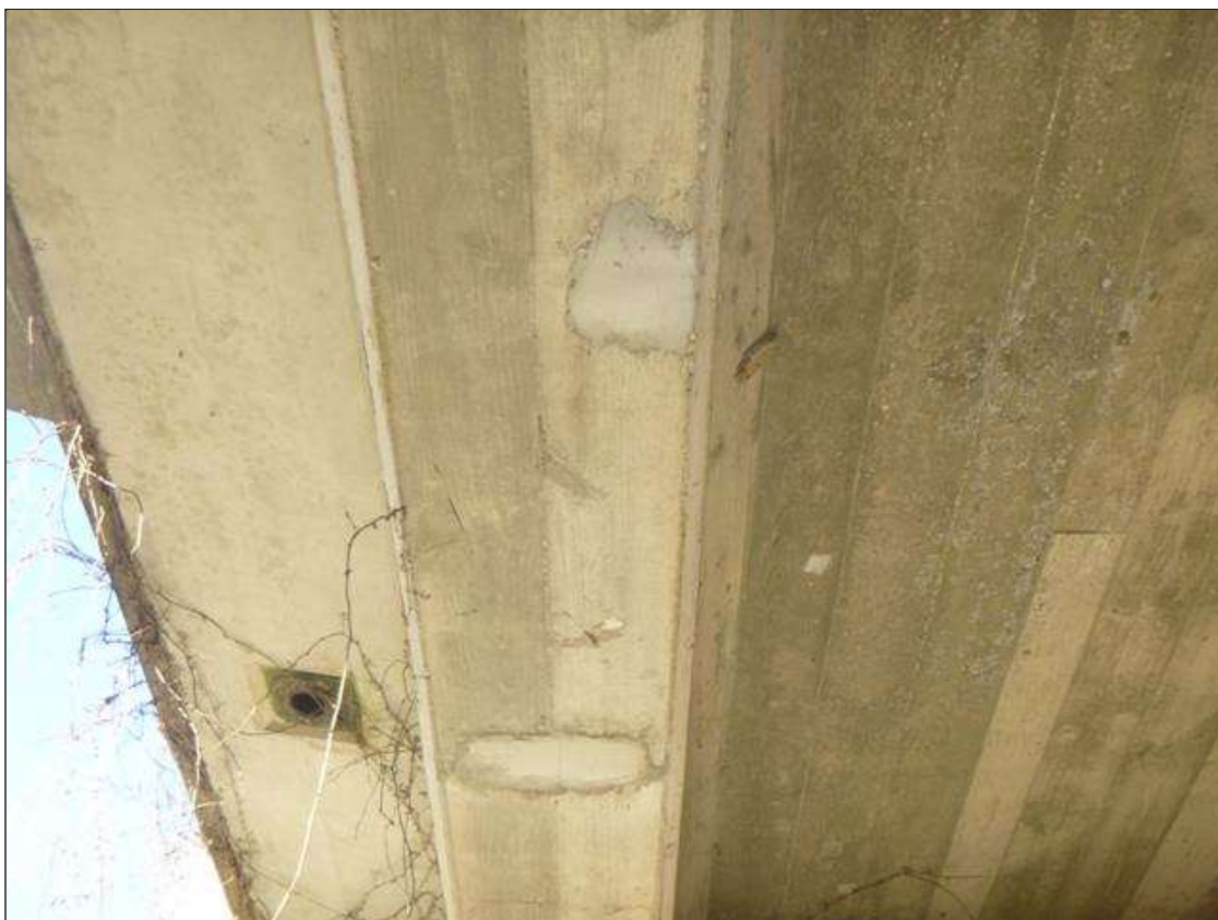
Span 3 Beam 1: 2- UP TO 9" X 6" CRACKED PATCHED AREA WITH UP TO 1/32" CRACKING ON UNDERSIDE OF BEAM 6' FROM ABUTMENT 2
