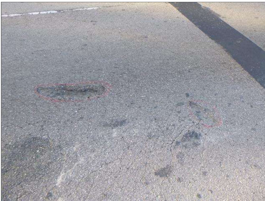
Span 1 Wearing Surface: 2- UP TO 20" X 6" X 1" POTHOLES, NEAR BENT 1 IN EAST LAST.
