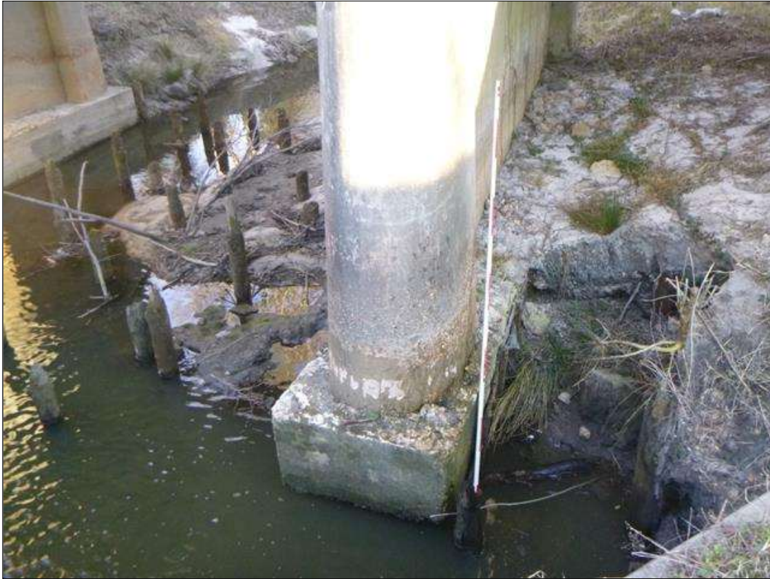
SCOUR: 35' X UP TO 15' X 9' SCOUR SOUTH EMBANKMENT AT PIER 1 UP TO 3' BELOW BOTTOM OF FOOTING AT PIER 1 SPAN 2 SIDE AND UPSTREAM END SPAN 1 SIDE WITH 6" OF UNDERMINING FULL WIDTH AT UPSTREAM END.
