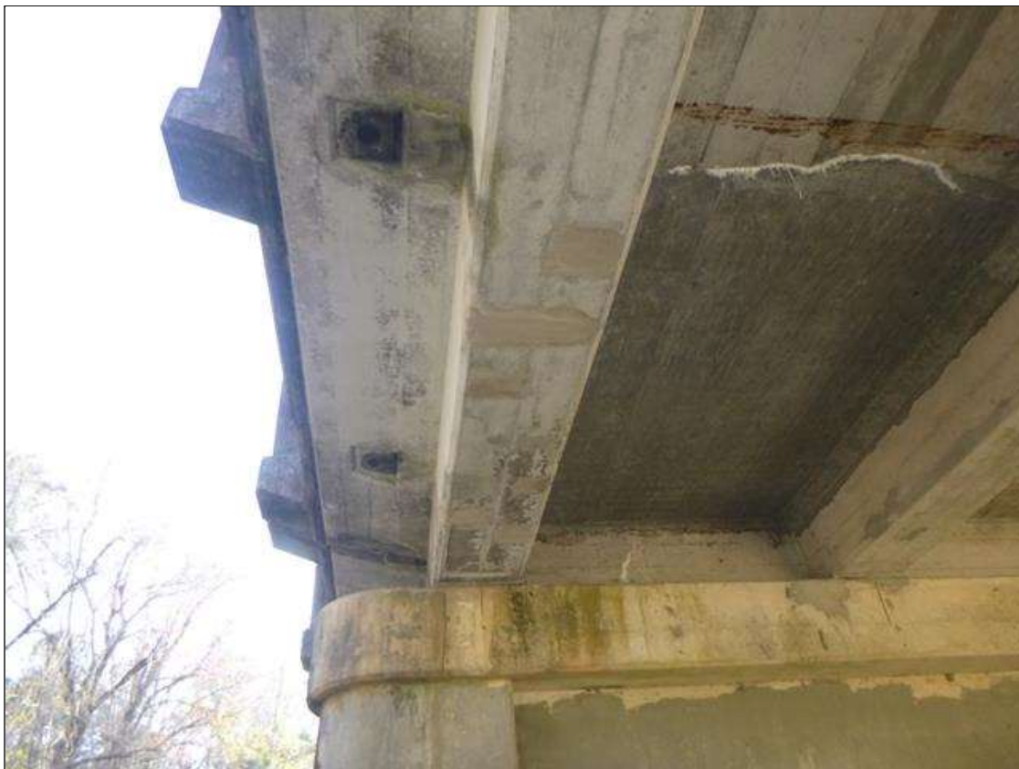
Span 3 Beam 4: SEVERAL SOUND PATCHED AREAS IN GIRDER 4 UNDERSIDE IN SPAN 3 STARTING AT PIER 2 (UP TO FULL WIDTH X 5" WIDE)
