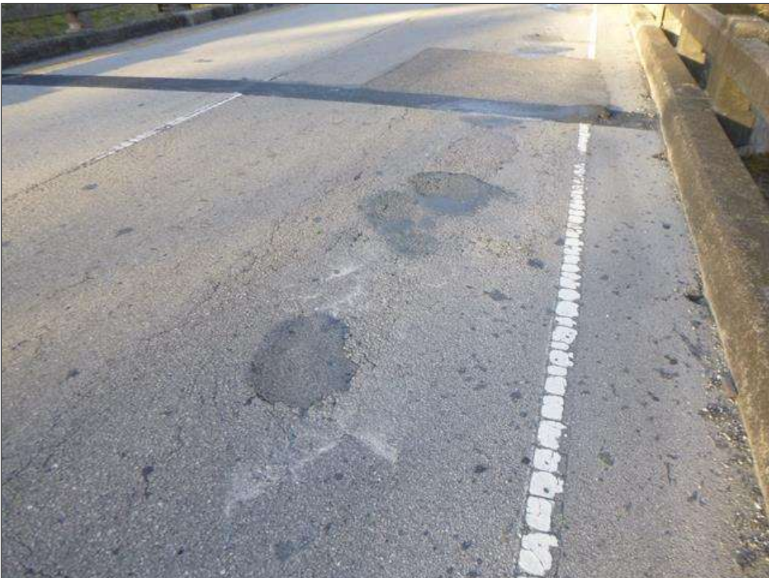
Span 2 Wearing Surface: A FEW SOUND PATCHED AREAS IN ASPHALT WEARING SURFACE LANE #2 RIGHT WHEEL PATH (10' FROM NORTH END) (UP TO 1.5' LONG X 2' WIDE)
