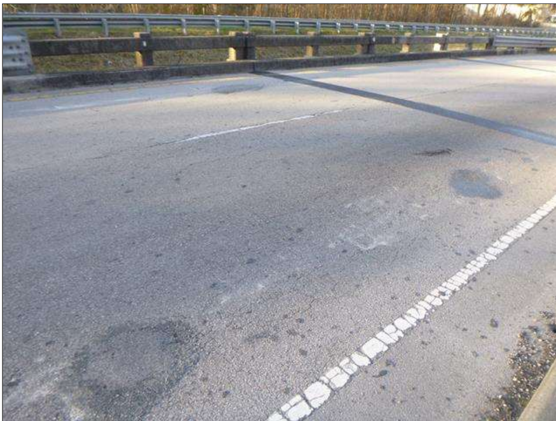
Span 1 Wearing Surface: 3- UP TO 3' X 1.5 SOUND PATCH IN ASPHALT WEARING SURFACE AT RANDOM THROUGHOUT.
