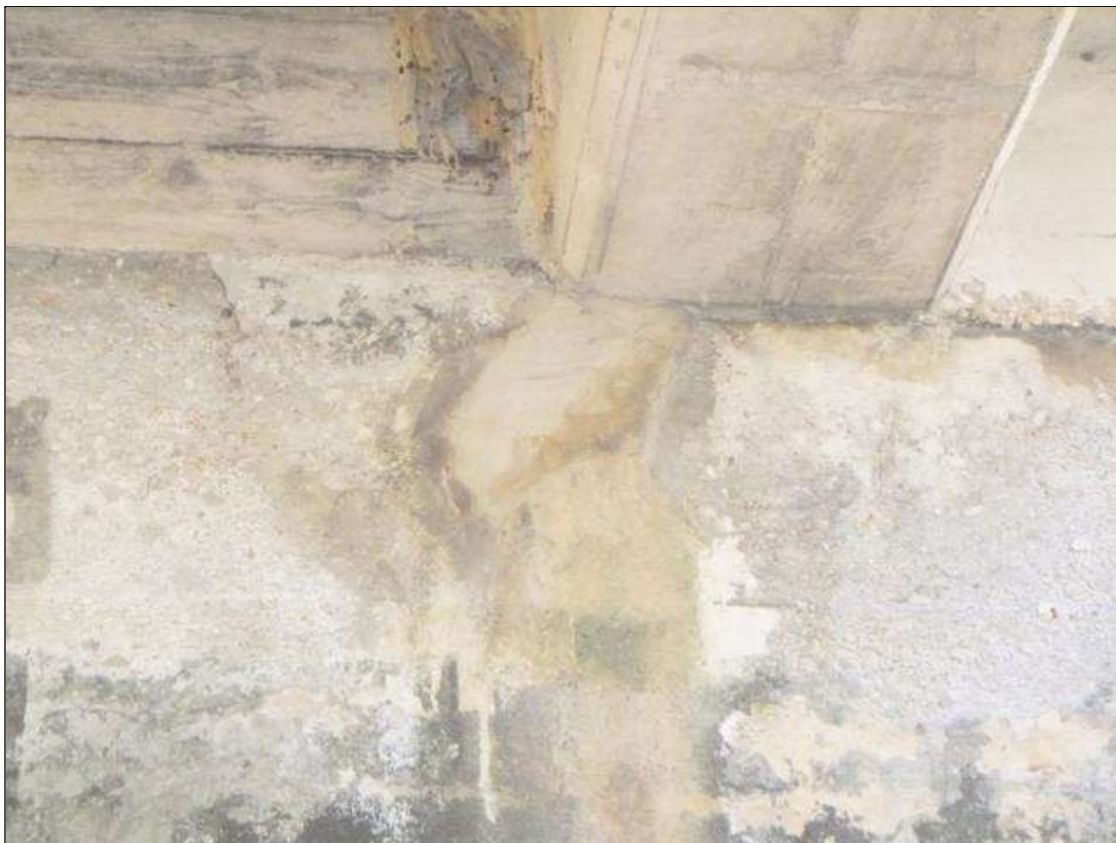
Abutment 2 Abutment: 1' X 1' CRACKED PATCHED AREA WITH UP TO 1/32" CRACKING WITH EFFLORESCENCE UNDER GIRDER 4.
