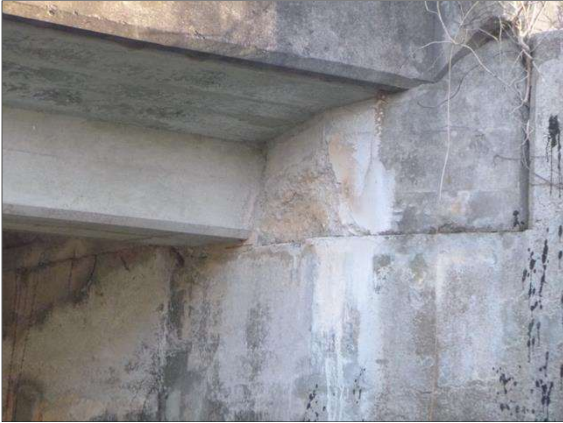
Abutment 1 Abutment: 2' X UP TO 14" X 5" SPALL UNDER WEST OVERHANG ADJACENT TO BEAM 1.
