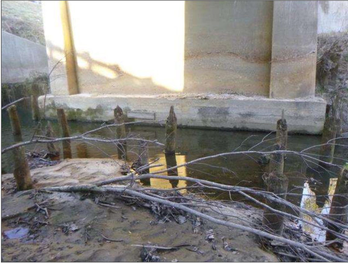
SCOUR: 35' X UP TO 15' X 9' SCOUR SOUTH EMBANKMENT AT PIER 1 UP TO 3' BELOW BOTTOM OF FOOTING AT PIER 1 SPAN 2 SIDE AND UPSTREAM END SPAN 1 SIDE WITH 6" OF UNDERMINING FULL WIDTH AT UPSTREAM END.
