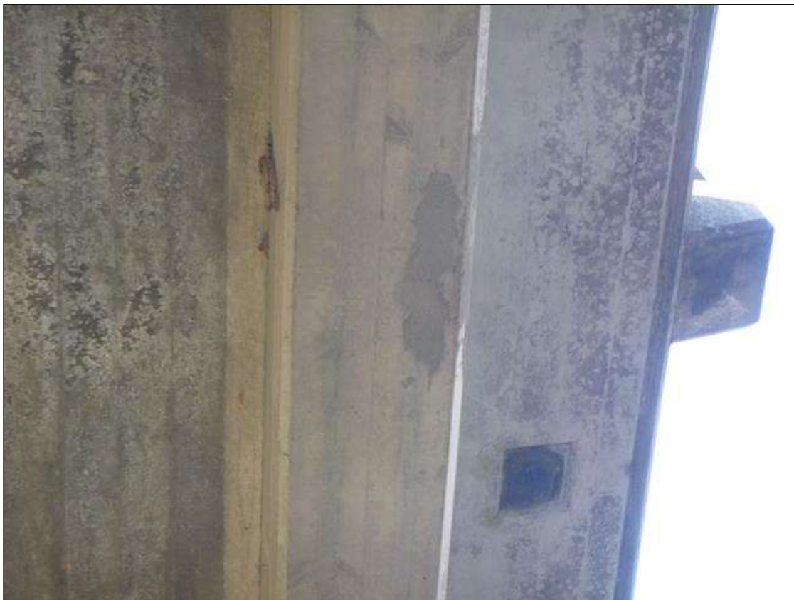
Span 2 Beam 4: 1.5' LONG X 6" WIDE SOUND PATCH ON UNDERSIDE OF BEAM 6' FROM PIER 1
