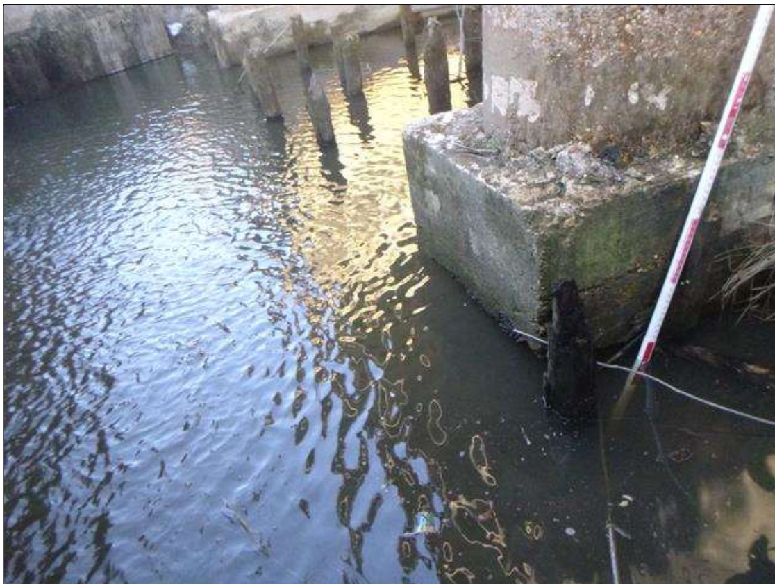
Bent 1 Footing: (PAR) SCOUR AROUND FOOTING ENTIRE LENGTH EXPOSING FOOTING WITH 6" OF UNDERMINING FULL WIDTH AT UPSTREAM END.
