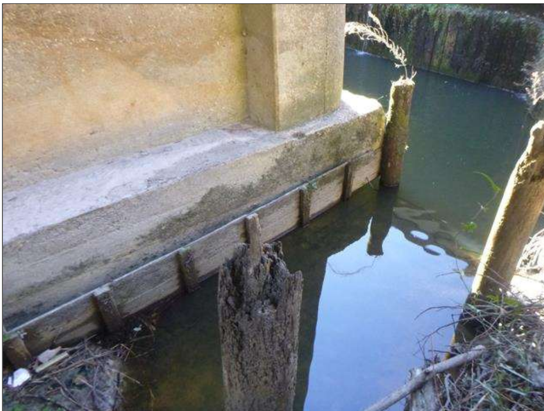
Bent 2 Footing: (PAR) SCOUR AROUND FOOTING FULL LENGTH EXPOSING FOOTING WITH 1' OF UNDERMINING FULL WIDTH AT UPSTREAM END
