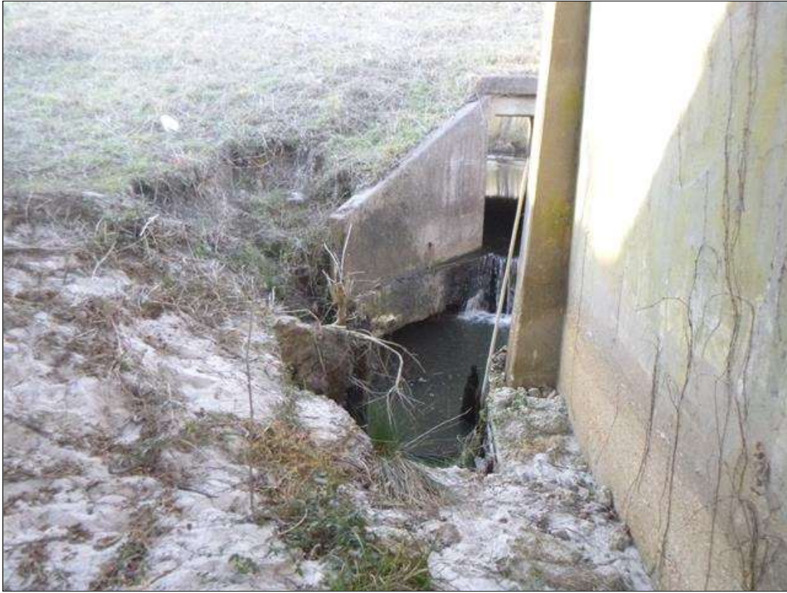
SCOUR: 35' X UP TO 15' X 9' SCOUR SOUTH EMBANKMENT AT PIER 1 UP TO 3' BELOW BOTTOM OF FOOTING AT PIER 1 SPAN 2 SIDE AND UPSTREAM END SPAN 1 SIDE WITH 6" OF UNDERMINING FULL WIDTH AT UPSTREAM END.
