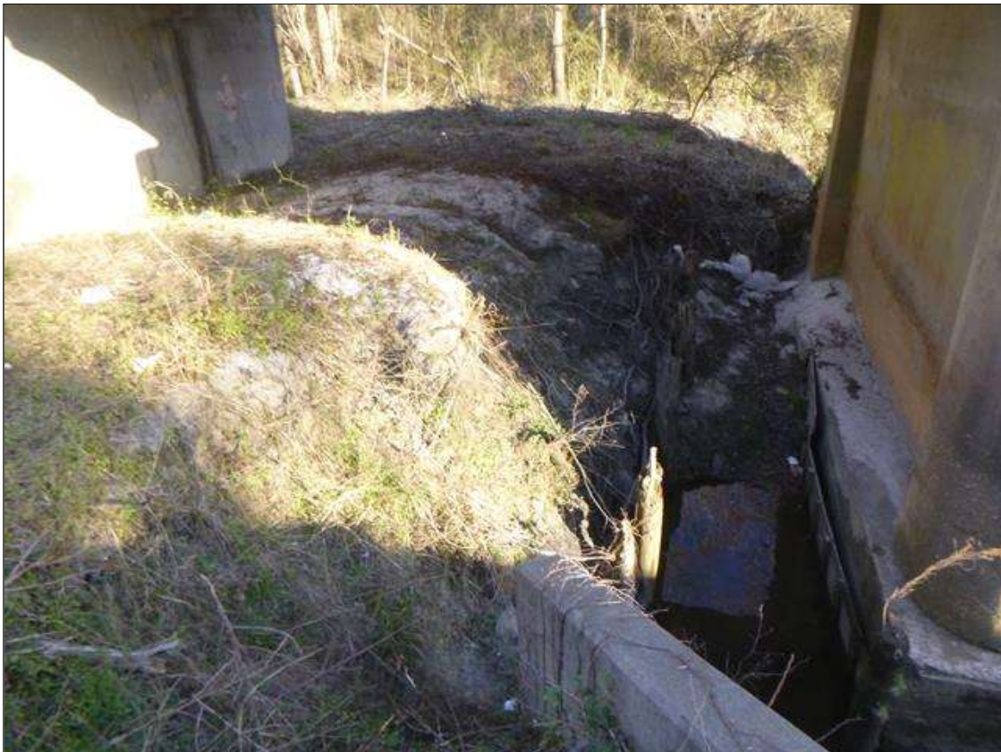
SCOUR: 15' X UP TO 40' X 6' DEEP SCOUR ALONG NORTH EMBANKMENT AT BENT 2 EXPOSING FOOTING AT PIER 2 FULL LENGTH WITH 1' OF UNDERMINING AT UPSTREAM END.
