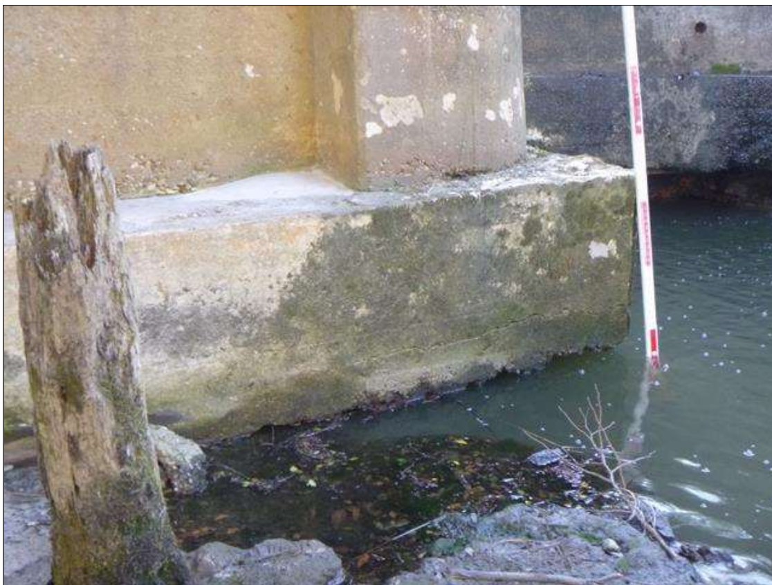
SCOUR: 35' X UP TO 15' X 9' SCOUR SOUTH EMBANKMENT AT PIER 1 UP TO 3' BELOW BOTTOM OF FOOTING AT PIER 1 SPAN 2 SIDE AND UPSTREAM END SPAN 1 SIDE WITH 6" OF UNDERMINING FULL WIDTH AT UPSTREAM END.
