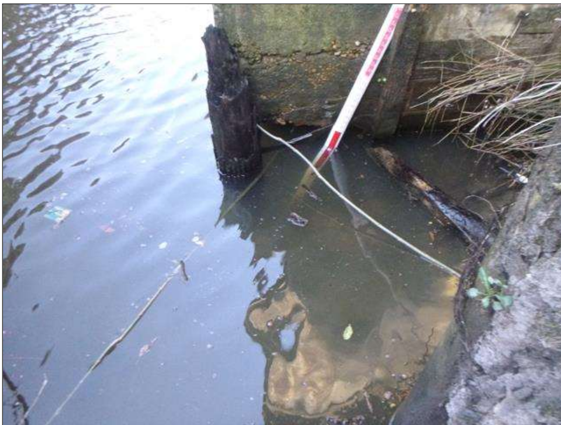
Bent 1 Footing: (PAR) SCOUR AROUND FOOTING ENTIRE LENGTH EXPOSING FOOTING WITH 6" OF UNDERMINING FULL WIDTH AT UPSTREAM END.
