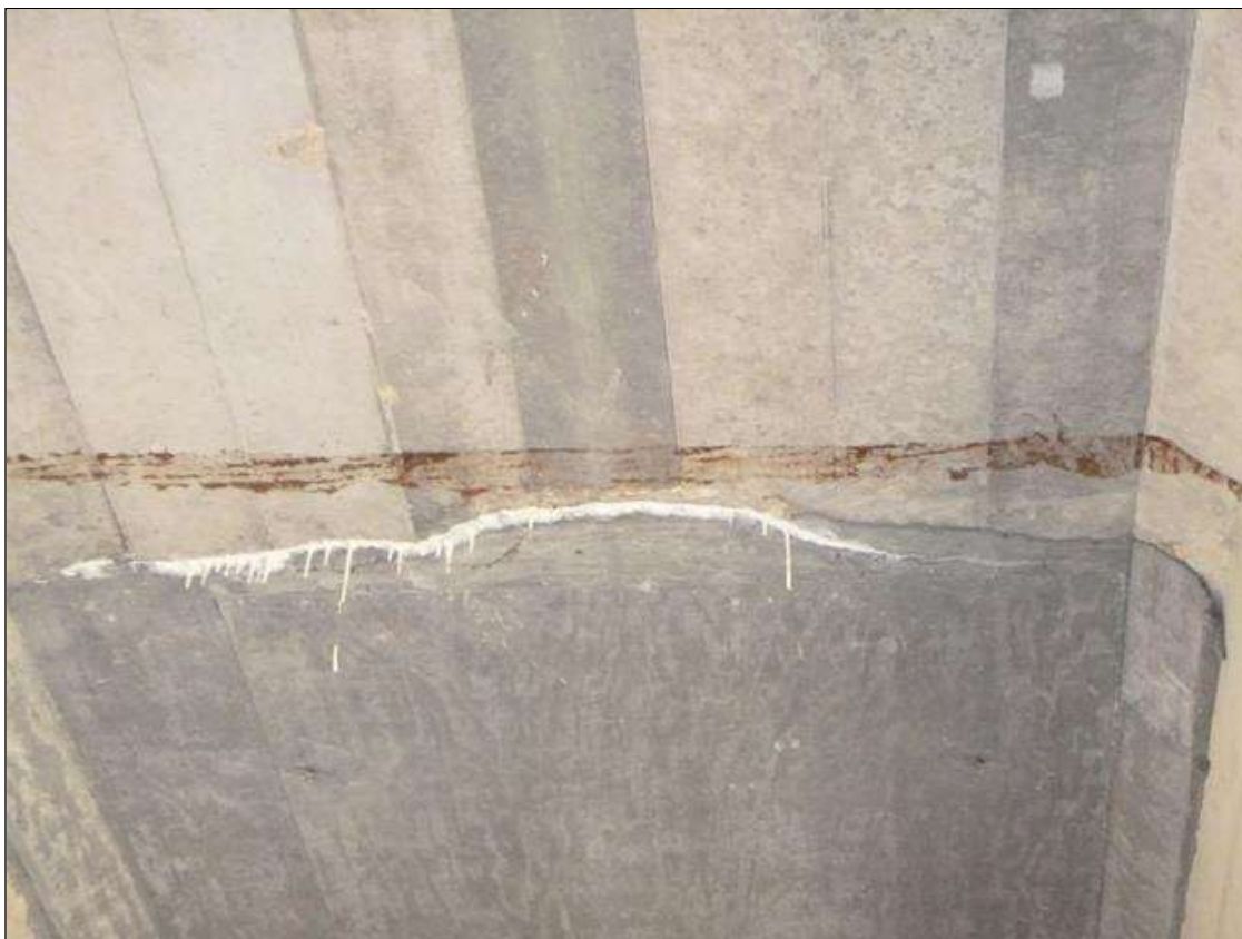
Span 3 Deck: HAIRLINE TRANSVERSE CRACK WITH EFFLORESCENCE BUILDUP IN SPAN 3 DECK UNDERSIDE IN BAY 3 AT END OF PATCHED AREA
