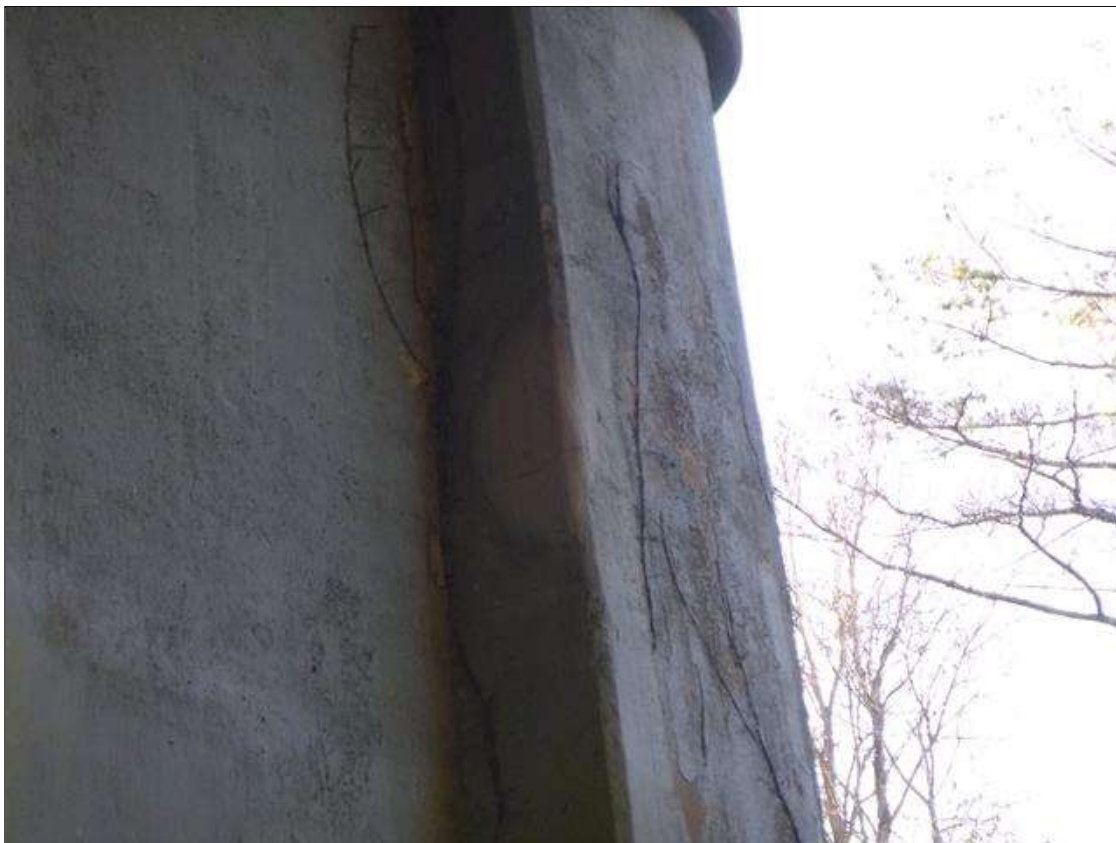
Bent 1 Pier 1: 15" X 9" CRACKED PATCHED AREA WITH UP TO 1/32" CEACKING IN NOSE PORTION NORTH FACE AT WEST END 5' FROM CAP
