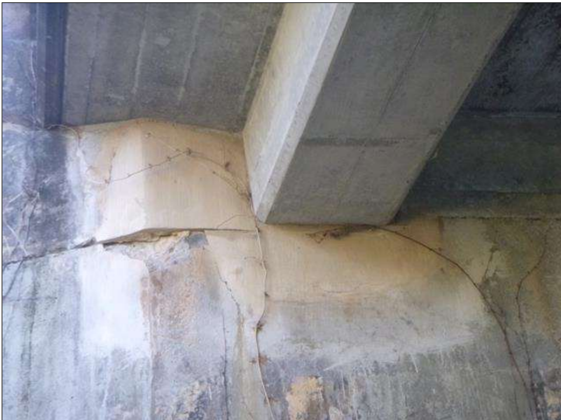
Abutment 1 Abutment: 3' WIDE X 1' HIGH SOUND PATCH AT TOP AT BEAM 4
