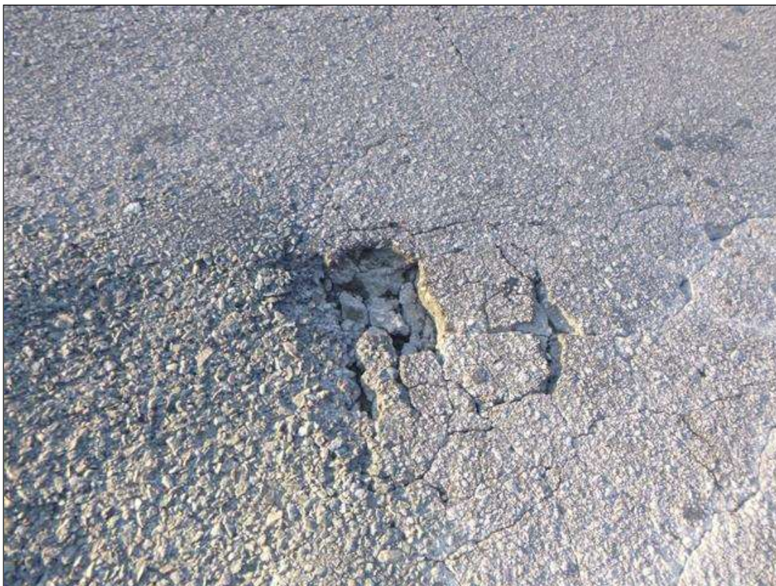
Span 3 Wearing Surface: 7" X 5" X 1" POTHOLE 5' FROM EAST BRIDGE RAIL AT MIDSPAN.
