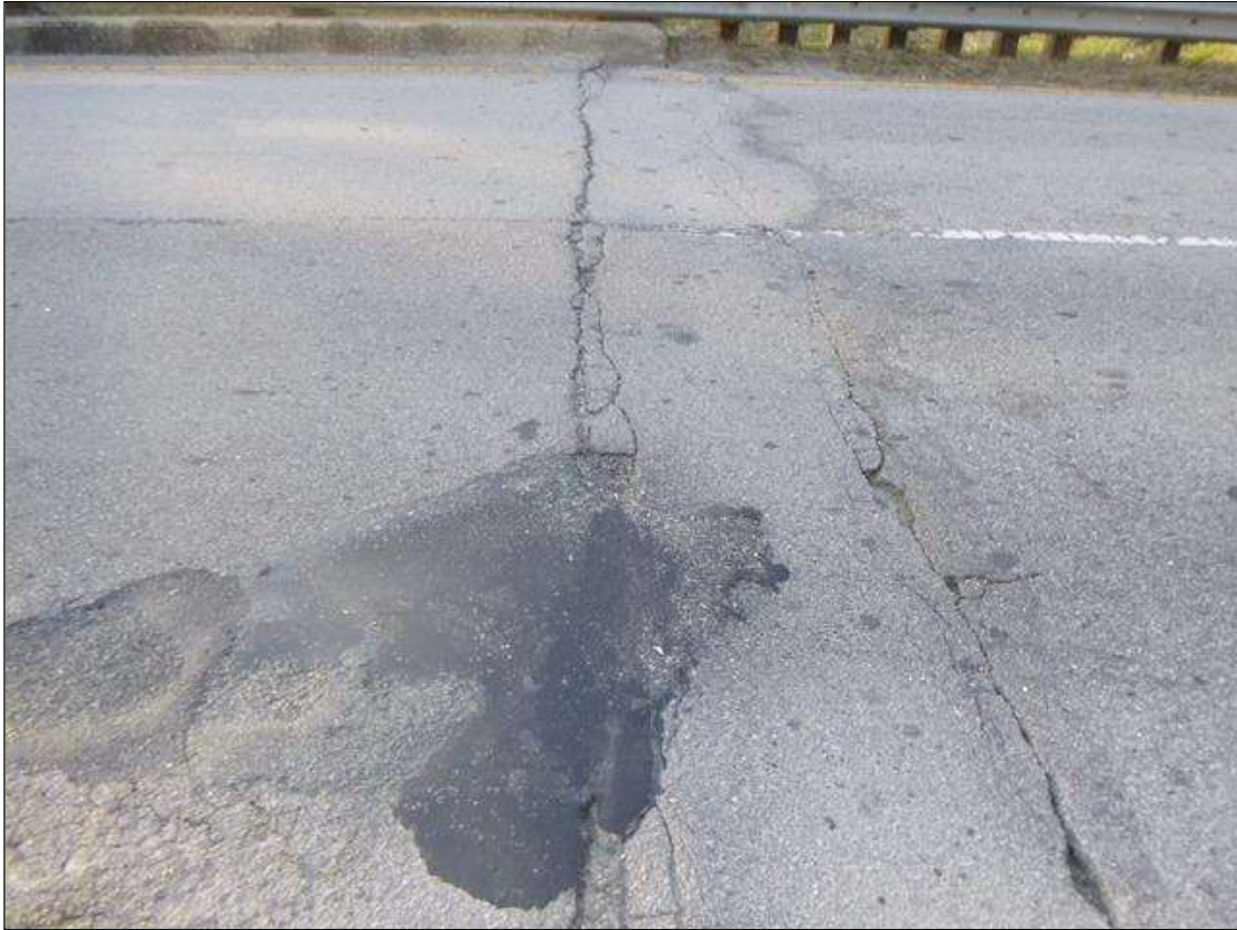
Span 3 Wearing Surface: TRANSVERSE CRACKING IN ASPHALT WEARING SURFACE OVER ABUTMENT 2 (UP TO 1/2" WIDE)
