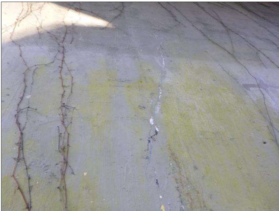
Bent 1 Pier 1: HAIRLINE VERTICAL CRACKING FULL HEIGHT AT CENTER POINT IN WALL ON SOUTH AND NORTH FACES
