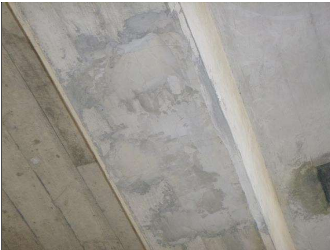
Span 3 Beam 4: CRACKED PATCHED AREA WITH UP TO 1/32" CRACKING IN GIRDER 4 UNDERSIDE IN SPAN 3, 5' FROM ABUTMENT 2 (2.5' LONG X 1.5' WIDE)
