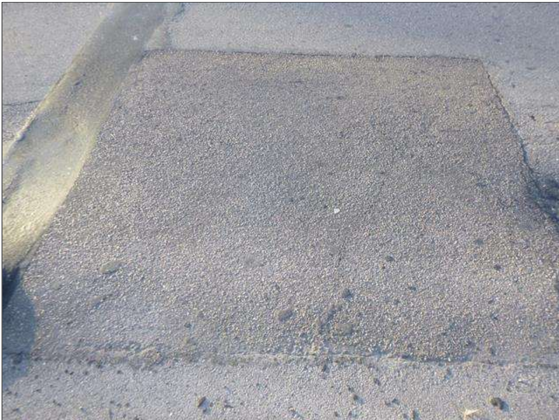
Span 3 Wearing Surface: 9' X 8' CRACKED PATCHED AREA WITH UP TO 1/4" CRACKING IN RIGHT LANE STARTING AT PIER 2
