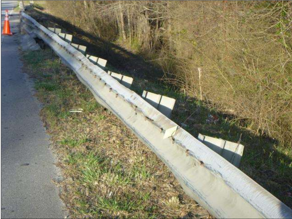
General Comments and Misc. Items: (PAR) 40' OF IMPACT DAMAGE, UP TO 1' DEFLECTION, GAUGES IN SOUTHEAST GUARDRAIL WITH 1 POST TO RAIL BOLT MISSING, 15' SOUTH OF BRIDGE.
