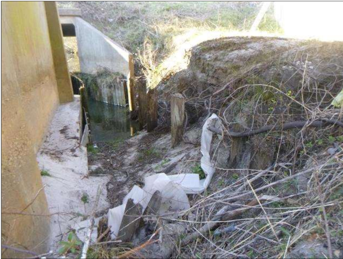
SCOUR: 15' X UP TO 40' X 6' DEEP SCOUR ALONG NORTH EMBANKMENT AT BENT 2 EXPOSING FOOTING AT PIER 2 FULL LENGTH WITH 1' OF UNDERMINING AT UPSTREAM END.
