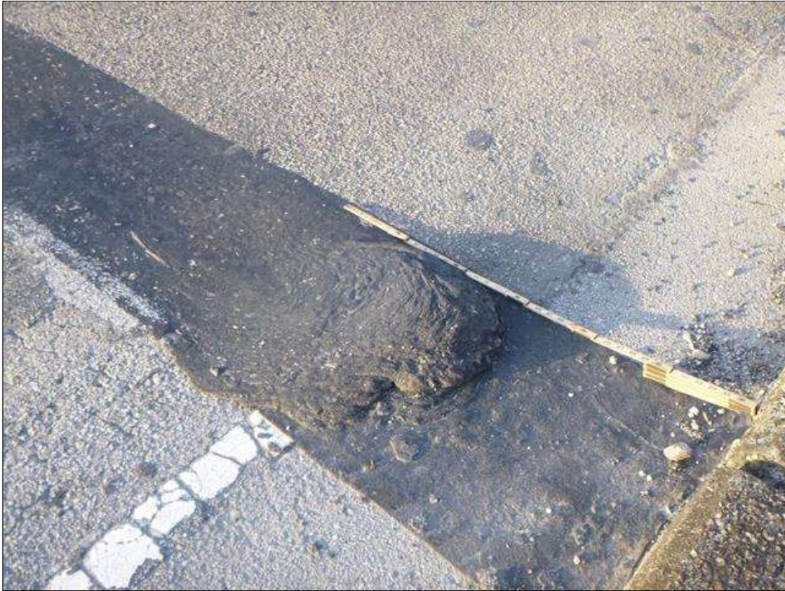
Span 2 Wearing Surface: UP TO 20" DIAMETER X 2" BUILDUP ON ASPHALT WEARING SURFACE OVER BENT 2, 2' FROM EAST BRIDGE RAIL.
