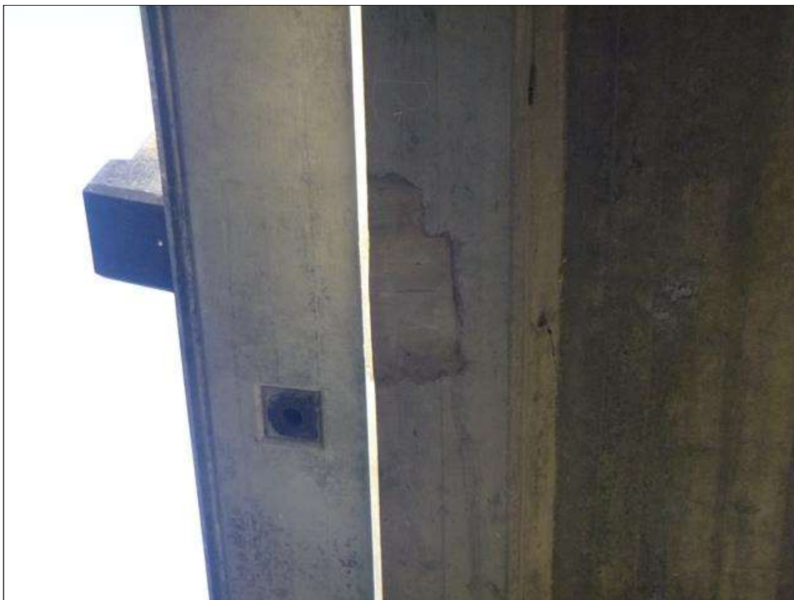
Span 2 Beam 1: SOUND PATCHED AREA 1.5' LONG X 8" WIDE IN GIRDER 1 UNDERSIDE IN SPAN 2, 6' FROM PIER 1.
