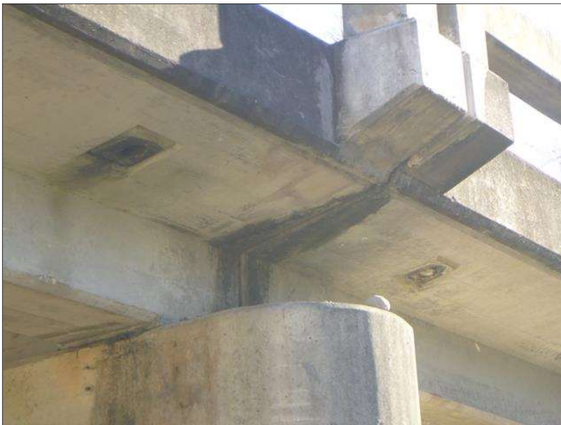
Span 3 Deck: SOUND PATCHED AREA WEST OVERHANG IN SPAN 3 BENT 2 (6" DIAMETER)
