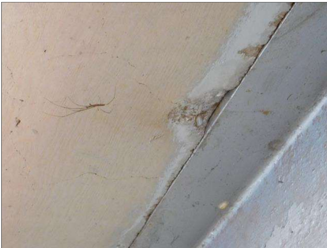
Span 2 Deck: 1" DIAMETER X 1/2" SPALL, WITH EXPOSED REINFORCING, DECK UNDERSIDE, BAY 7, ADJACENT TO BEAM 8, NEAR MID-SPAN.
