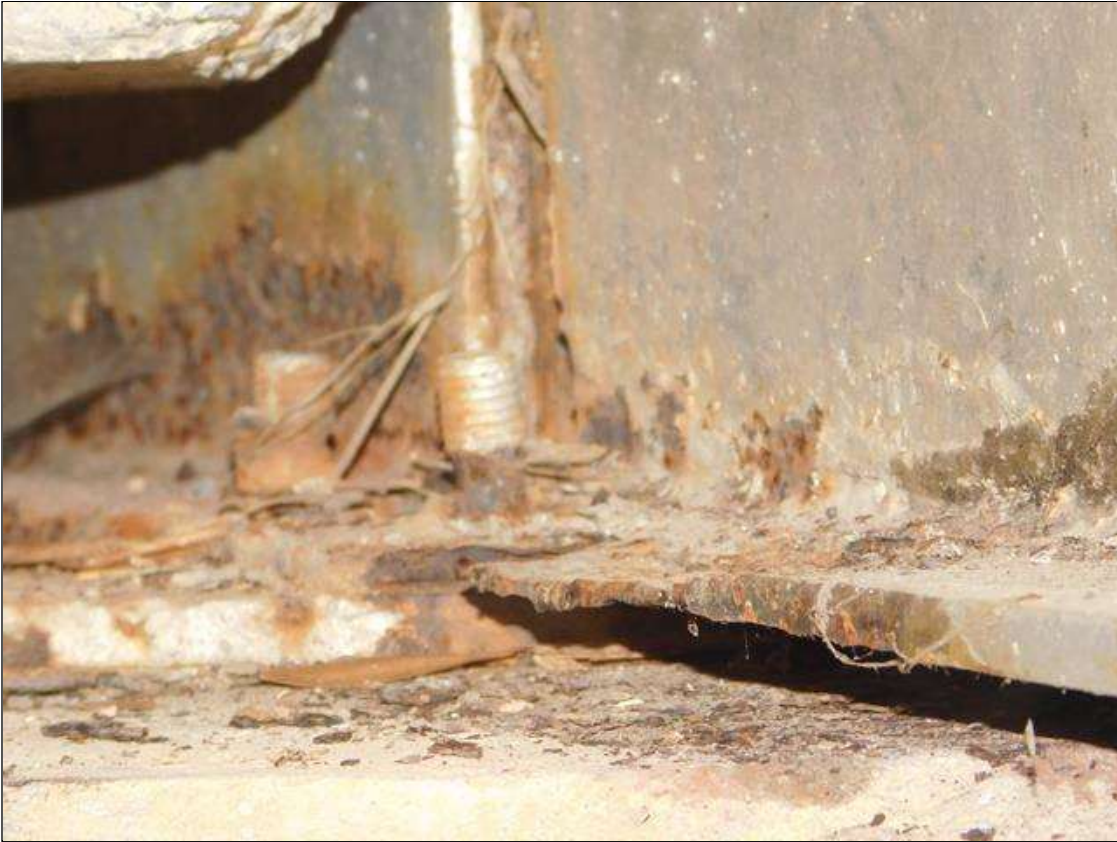
Span 1 Beam 8: 18" OF RUST SCALE, BOTTOM FLANGE, UP TO 5" IN THE WEB, 1/4" REMAINING IN THE BOTTOM FLANGE. WITH A 2" DIAMETER AREA WITH 100% SECTION LOSS AT BENT 1. A "PAR" HAS BEEN ISSUED FOR THIS CONDITION.
