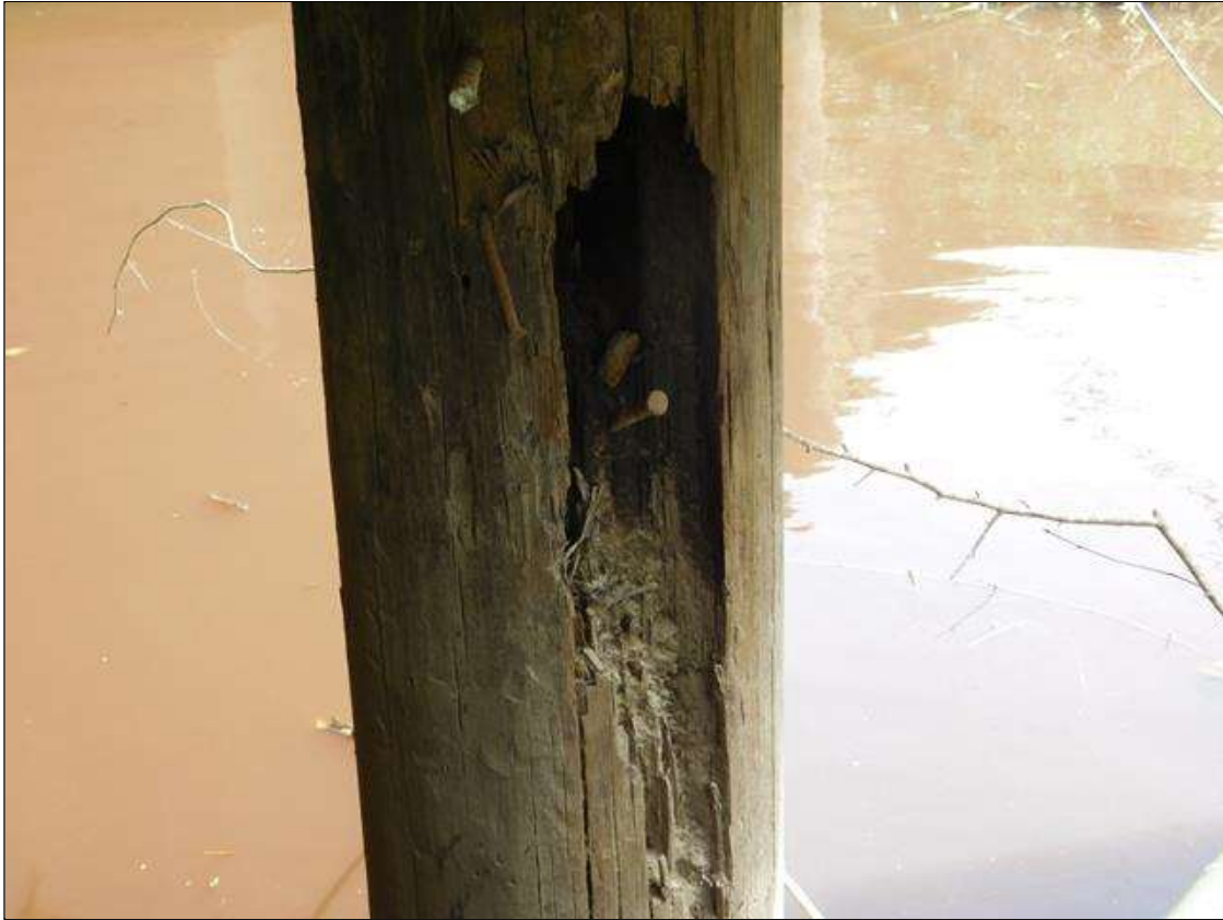
Bent 1 Pile 5: at Southeast quadrant from cap down 3ft, decay [3ft x 7in x up to 9in deep] crutch bent installed at both sides of bent 1
