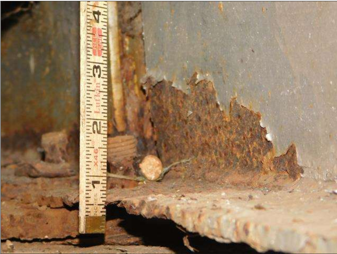
Span 1 Beam 2: 6" OF RUST SCALE, BOTTOM FLANGE, UP TO 2" IN THE WEB, WITH 1/16" REMAINING IN THE BOTTOM FLANGE, AT BENT 1. A "PAR" HAS BEEN ISSUED FOR THIS CONDITION.
