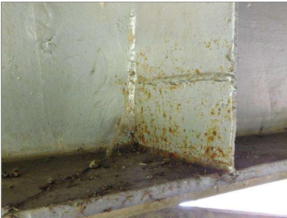
Span 1 Crutch Bent 1 Cap 1: 7" X 2" AREA OF RUST SCALE, WITH 1" X 1" HOLE, SOUTH BEARING STIFFENER, 4' WEST OF PILE 2. / THIS AREA HAS BEEN REPAIRED
