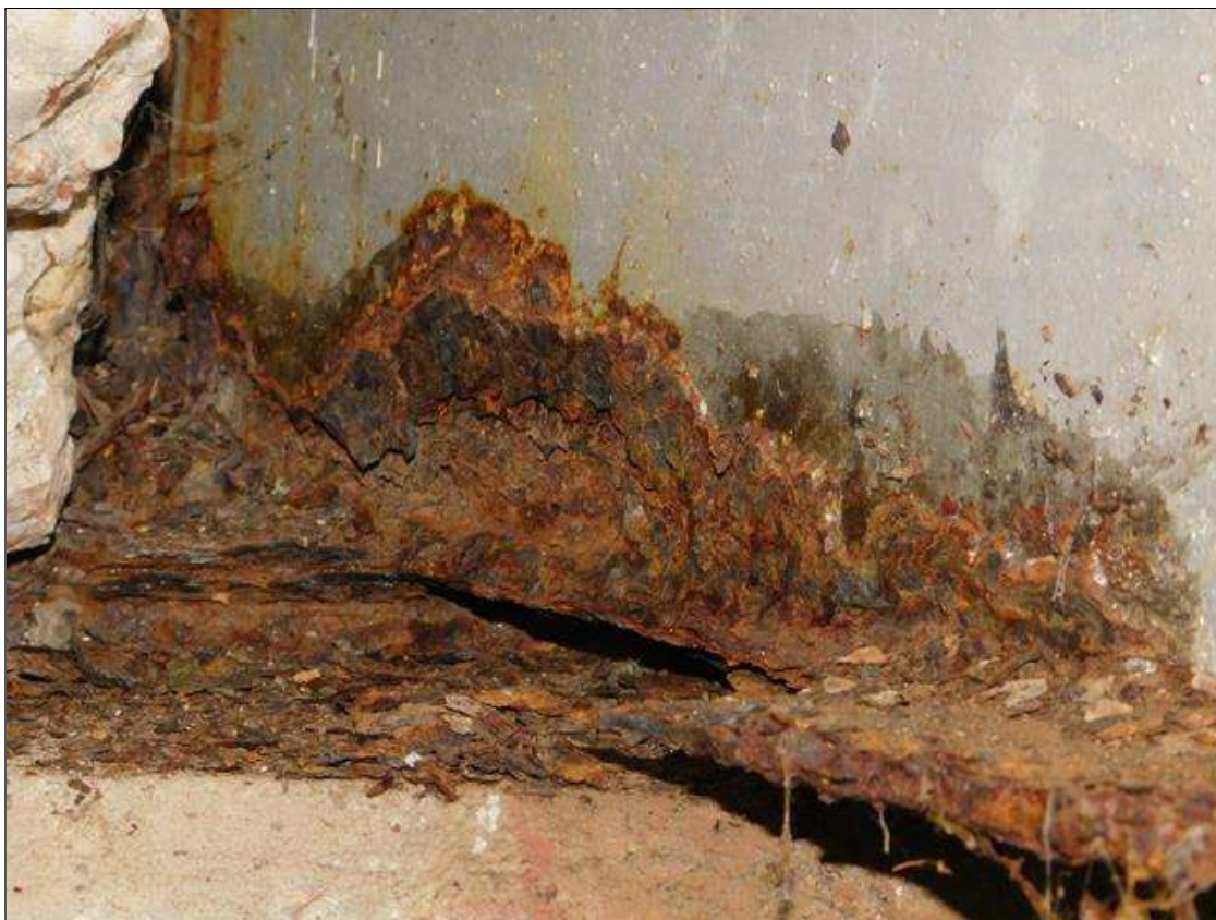
Span 2 Beam 1: RIGHT WEB AND BOTTOM FLANGE OVER BENT 1. HAS A 10" x 3" AREA OF 100% SECTION LOSS. A "PAR" HAS BEEN ISSUED FOR THIS CONDITION.
