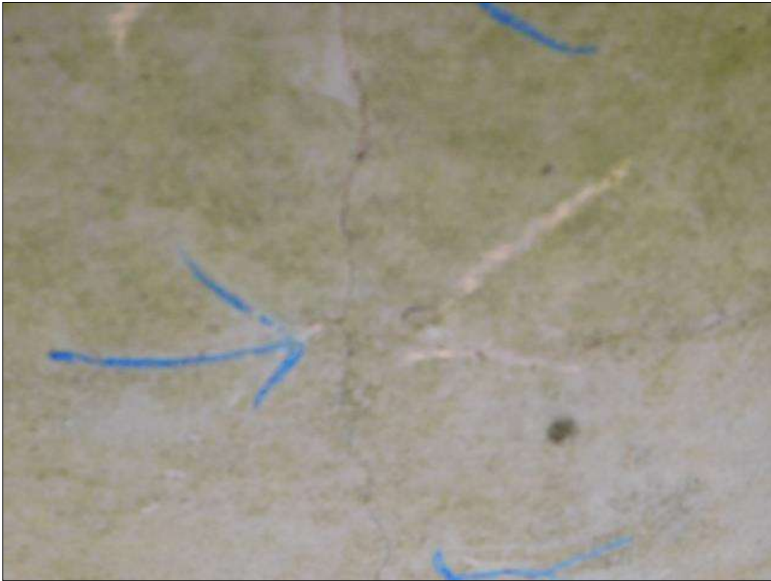
Span 1 Deck: along underside of deck, multiple transverse cracks [up to 8ft x 0.02in]
