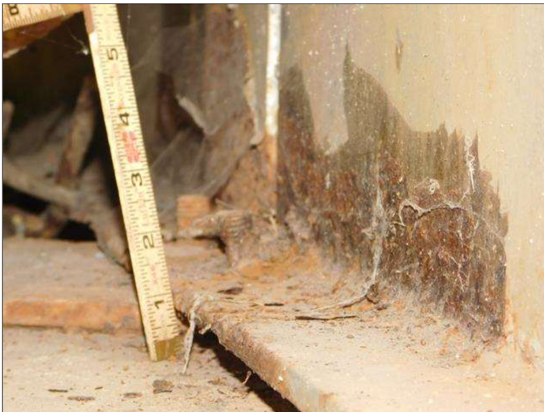
Span 2 Beam 6: 3' OF RUST SCALE, TOP AND BOTTOM FLANGE, UP TO 3" IN THE WEB, WITH 1/4" REMAINING IN THE BOTTOM FLANGE, AT BENT 1. BOTTOM FLANGE HAS A 1" DIAMETER HOLE. A "PAR" HAS BEEN ISSUED FOR THIS CONDITION.
