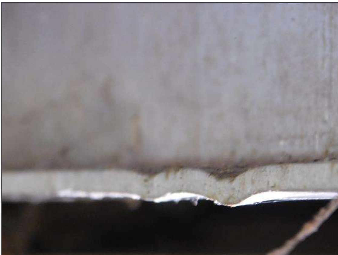
Span 1 Beam 6: West bottom flange near Mid-Span, distortion [6in x 1/4in]
