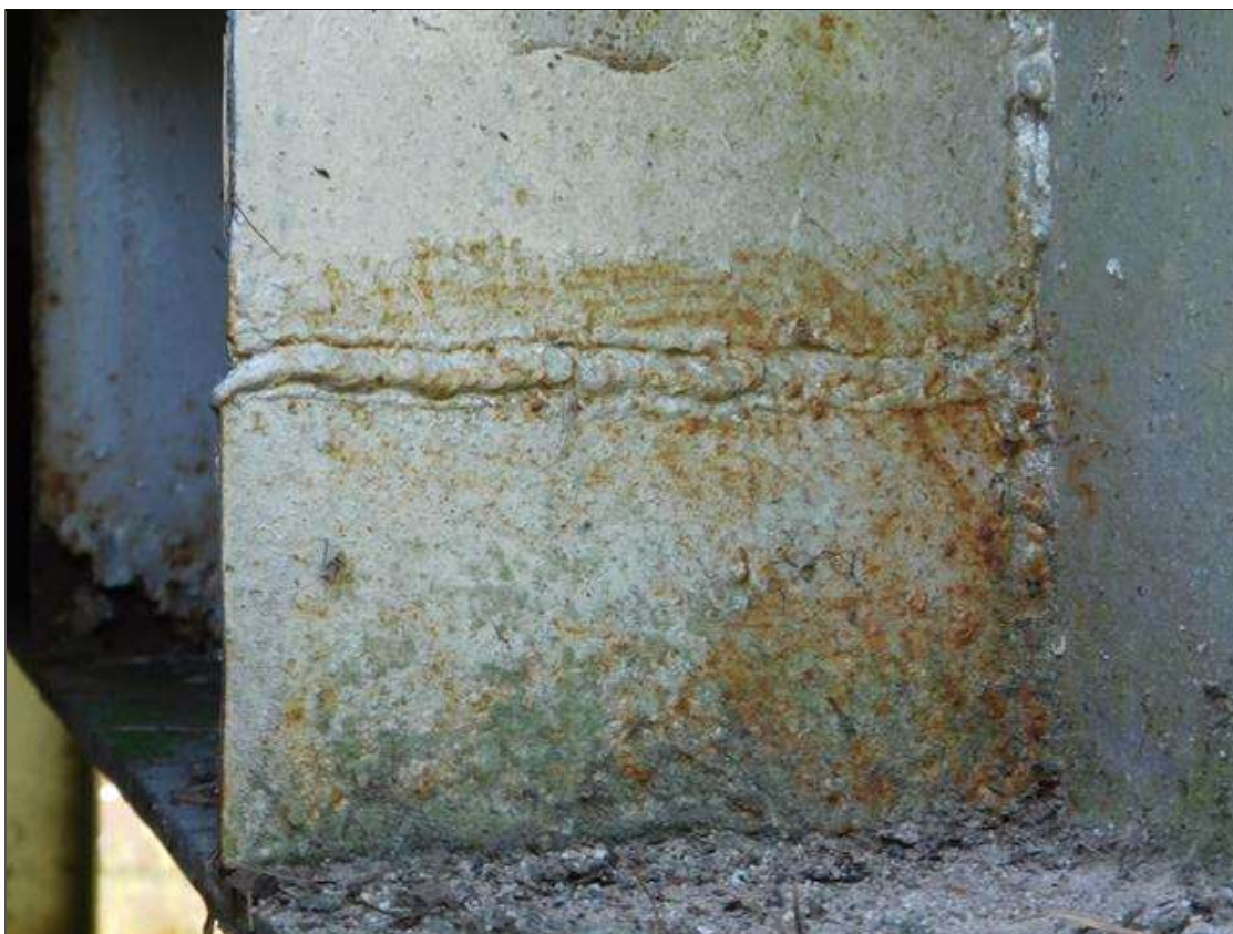
Span 1 Crutch Bent 1 Cap 1: 7" X 3" AREA OF RUST SCALE, WITH 2" DIAMETER HOLE, NORTH BEARING STIFFENER, ABOVE PILE 1. / THIS AREA HAS BEEN REPAIRED
