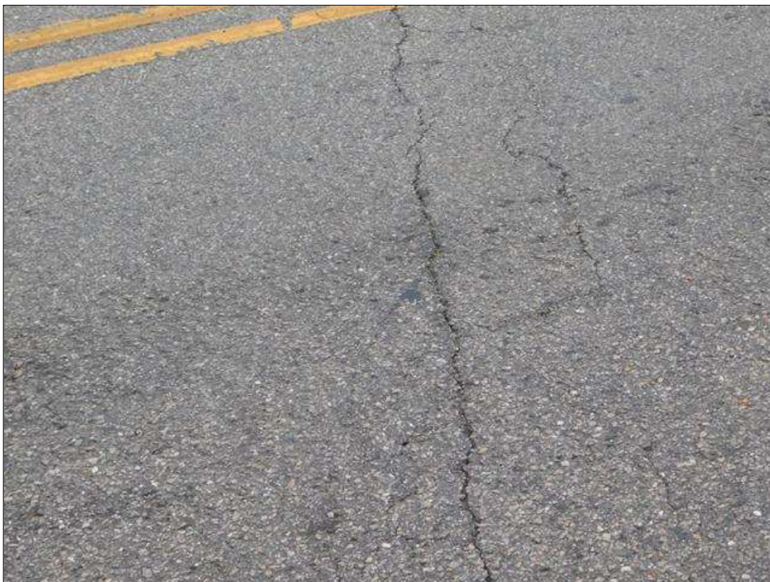
Span 1 Wearing Surface: at End Bent 1, transverse crack [full width x 1/8in]
