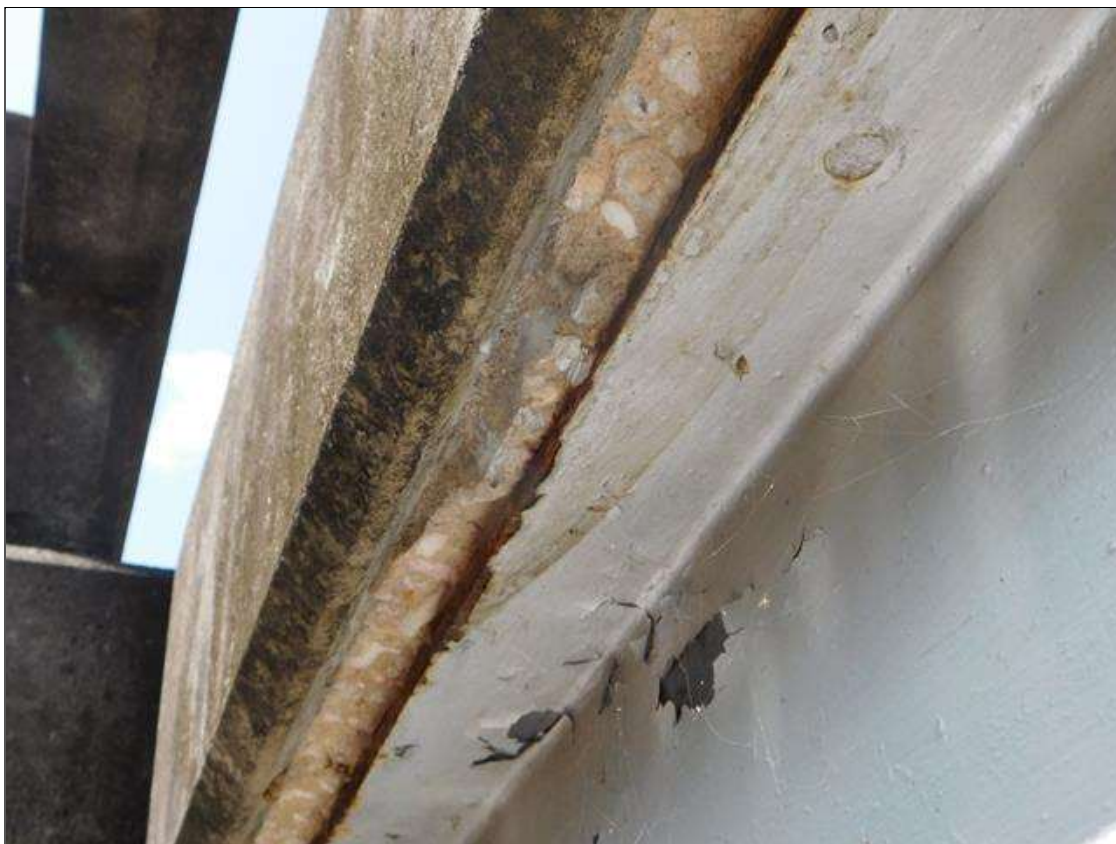
Span 2 Deck: 10' X UP TO 2" X 1" SPALL, DECK UNDERSIDE, RIGHT OVERHANG, BEGINNING AT BENT 1.
