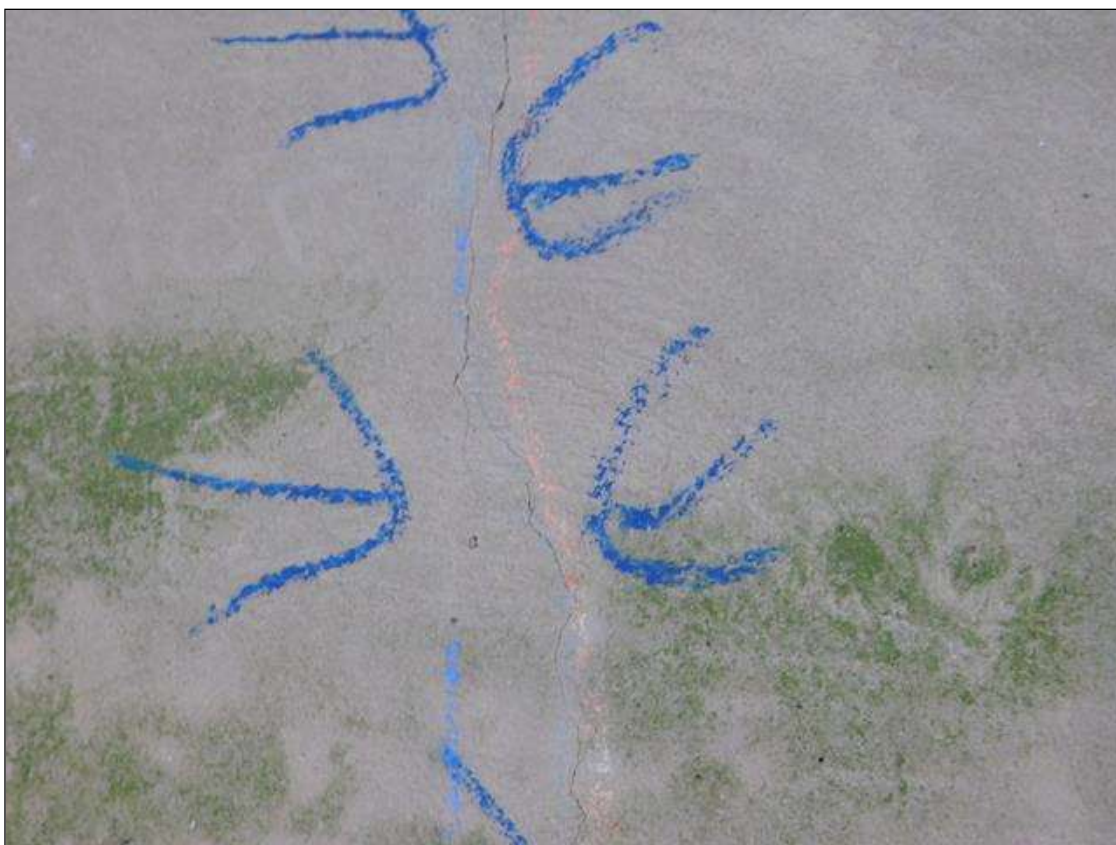
End Bent 1 Cap 1: (8) UP TO 16" X 1/16" VERTICAL CRACKS, NORTH FACE, AT RANDOM THROUGHOUT.
