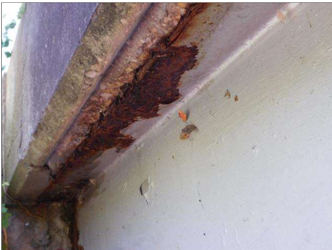
Span 2 Beam 1: at near and far ends, surface corrosion [2ft x up to full height x full width]
