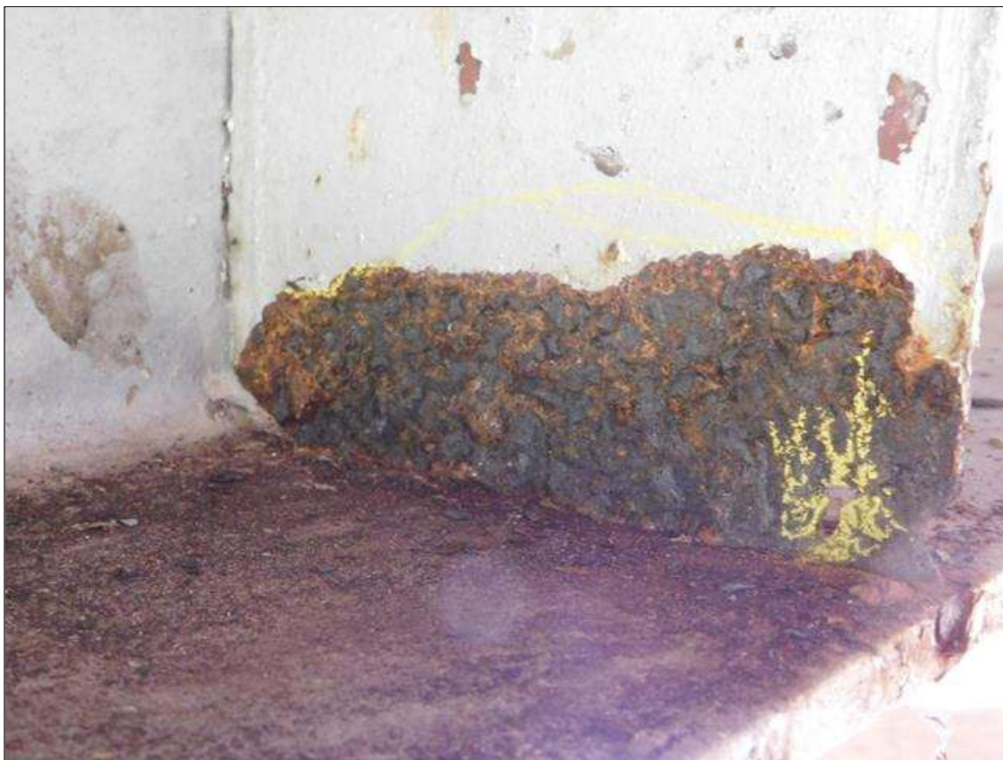
Span 1 Crutch Bent 1 Cap 1: BEARING STIFFNER UNDER BEAM 5. HAS A 7" x 2" AREA OF SECTION LOSS DOWN TO A KNIFE EDGE REMAINING. WITH A 1/2" DIAMETER HOLE. A "PAR" HAS BEEN ISSUED FOR THIS CONDITION.
