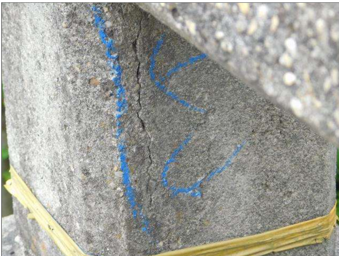
Span 1 Left Bridge Rail: NORTH FACE OF POST 1 HAS A 1/16" WIDE x 8" HIGH VERTICAL CRACK.
