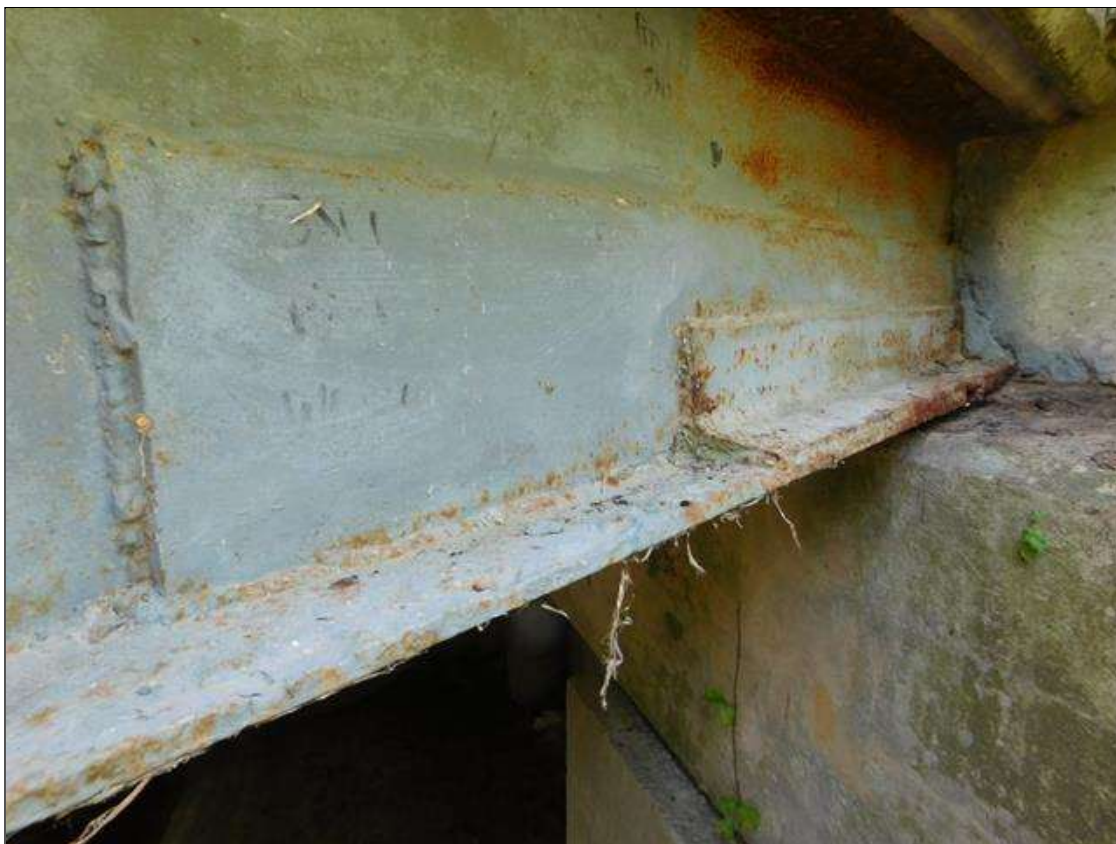
Span 1 Beam 1: 1' OF RUST SCALE, BOTTOM FLANGE, WITH 3/8" REMAINING IN THE BOTTOM FLANGE, WITH 3' X 7" WEB PLATE AND 2' X 3" REPAIR ANGLE ON WEST FACE, AT END BENT 1.
