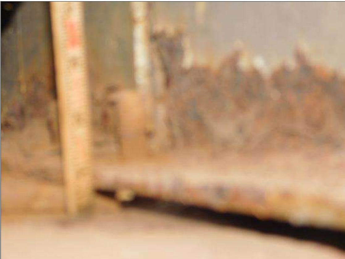
Span 1 Beam 3: 1' OF RUST SCALE, BOTTOM FLANGE, UP TO 3" IN THE WEB, WITH 1/4" REMAINING IN THE BOTTOM FLANGE, AT BENT 1. A "PAR" HAS BEEN ISSUED FOR THIS CONDITION.
