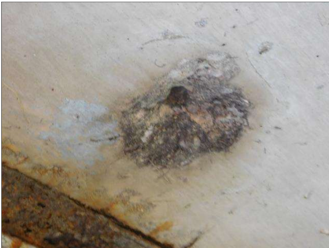
Span 2 Deck: 4" DIAMETER X 1" SPALL, WITH EXPOSED REINFORCING, DECK UNDERSIDE, BAY 1, 3' FROM END BENT 2.
