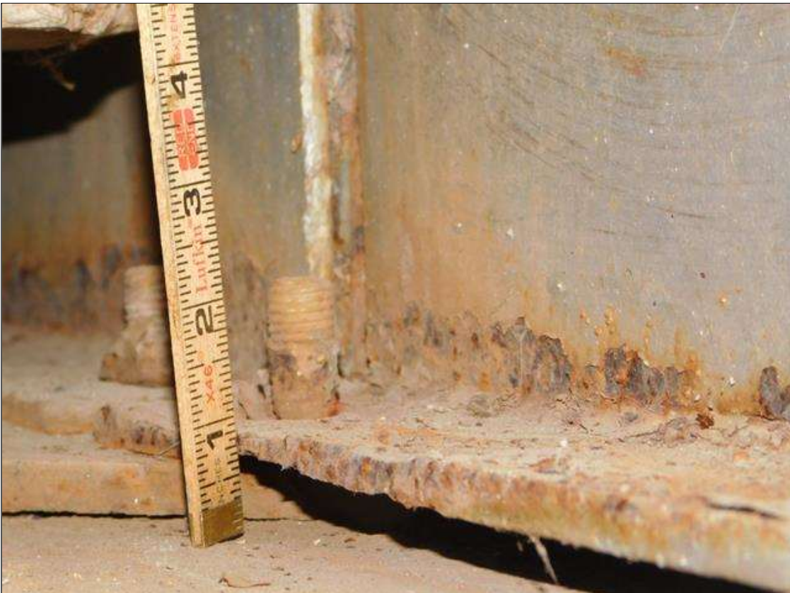
Span 1 Beam 5: 18" OF RUST SCALE, BOTTOM FLANGE, UP TO 4" IN THE WEB, WITH 1/4" REMAINING IN THE BOTTOM FLANGE, AT BENT 1. A "PAR" HAS BEEN ISSUED FOR THIS CONDITION.
