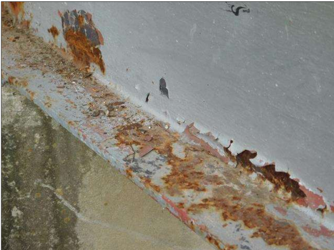
Span 1 Beam 11: 6" OF RUST SCALE, BOTTOM FLANGE, UP TO 2" IN THE WEB, AT END BENT 1.
