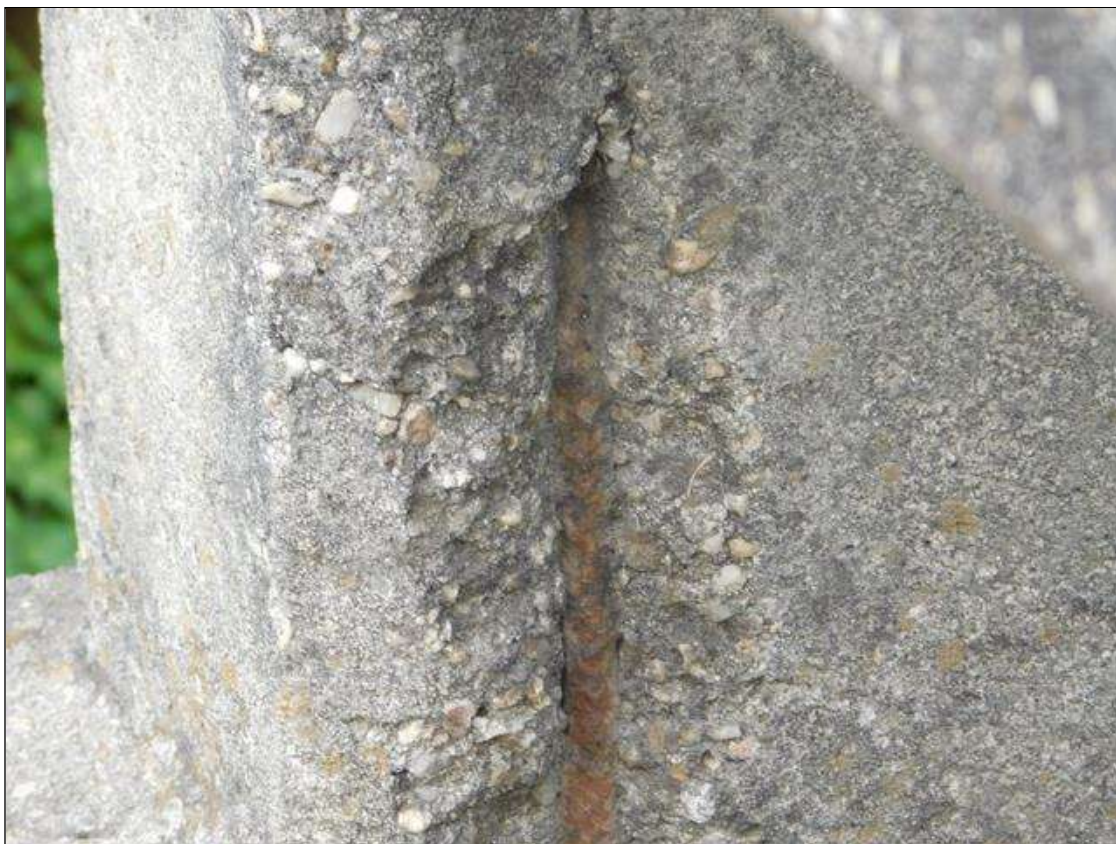
Span 1 Left Bridge Rail: at base of rail post 2, spall [8in x 2in x 3/4in deep] with exposed rusted reinforcing no section loss noted
