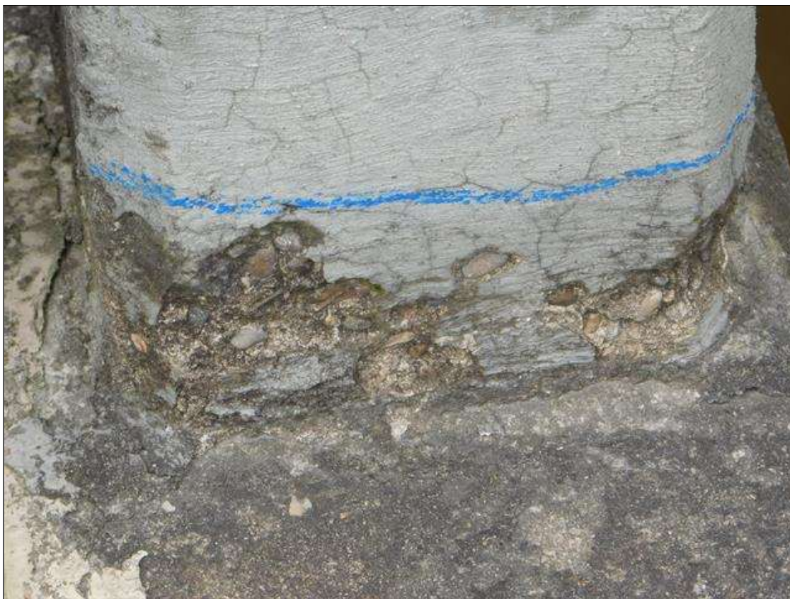
Span 2 Left Bridge Rail: LEFT RAIL POST 1 EAST FACE NEAR BOTTOM. HAS A 10" x 4" x 1/4" DEEP SPALL.
