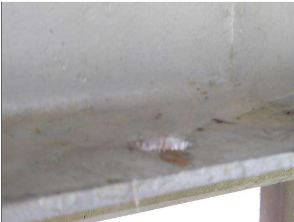
Span 2 Crutch Bent 2 Cap 1: 1" DIAMETER HOLE, BOTTOM FLANGE, 1' WEST OF PILE 2.
