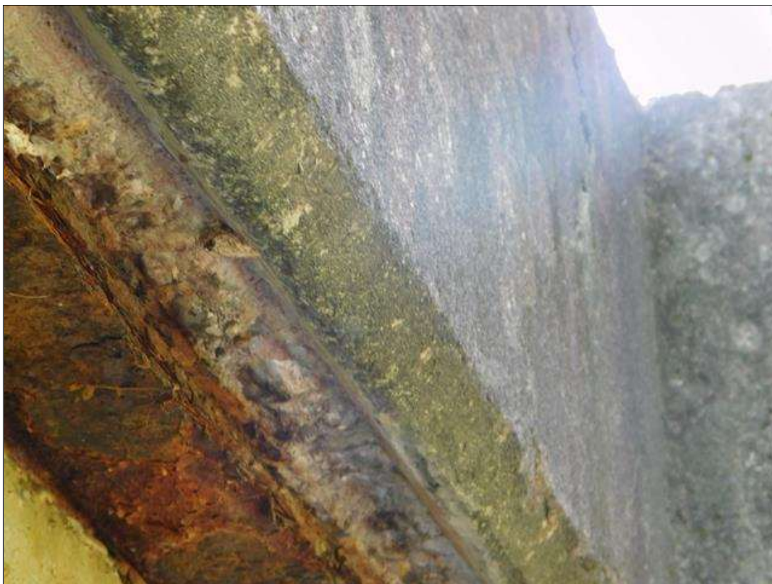
Span 2 Deck: 3' X 2" X 1" SPALL, DECK UNDERSIDE, LEFT OVERHANG, AT BENT 1.
