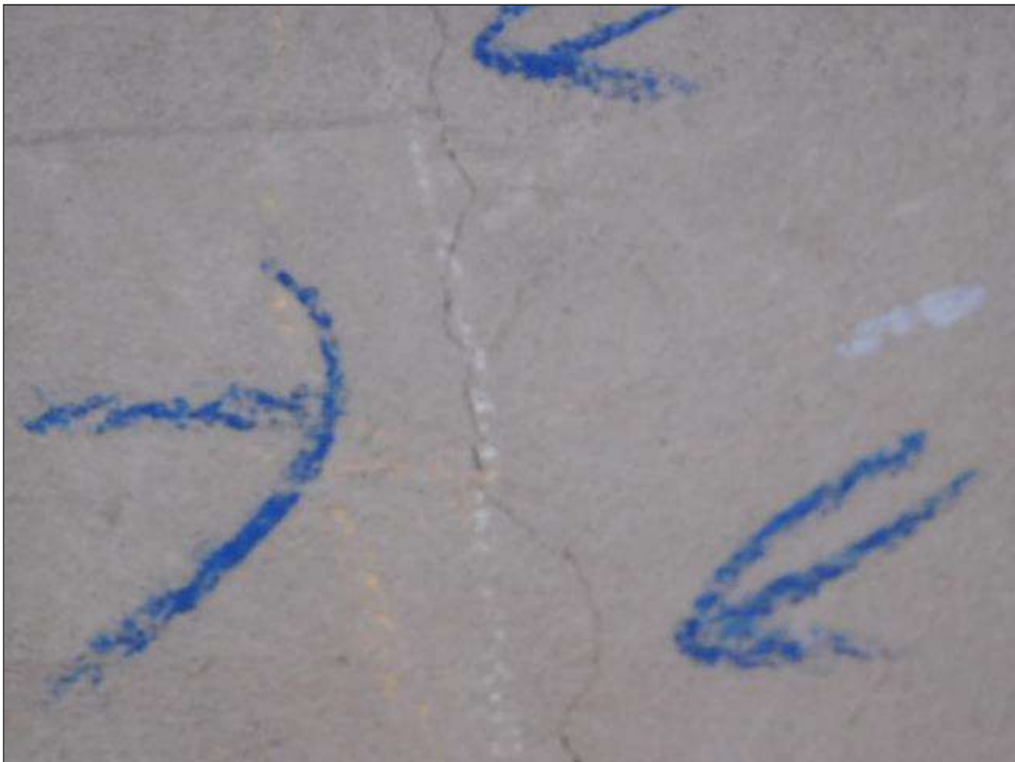
End Bent 2 Cap 1: along length of cap, multiple vertical cracks [1ft x 0.02in]
