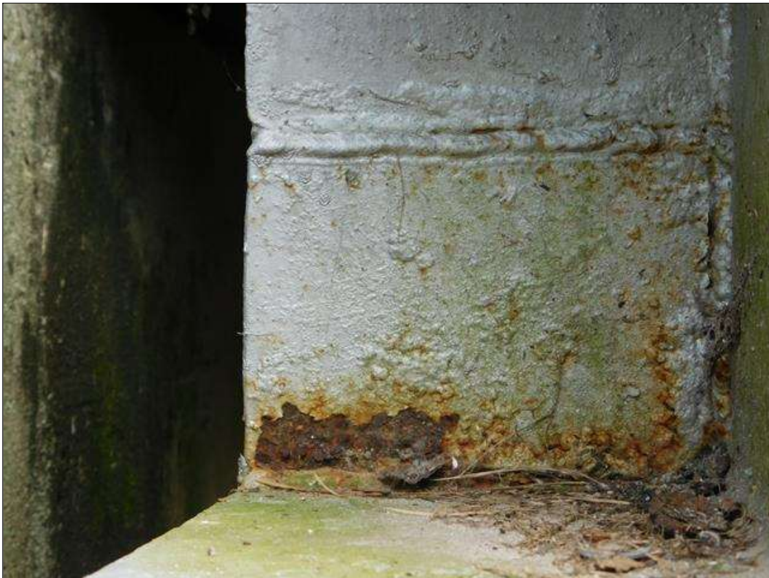
Span 2 Crutch Bent 2 Cap 1: 7" X 3" AREA OF RUST SCALE, WITH 3" X 2" HOLE, SOUTH BEARING STIFFENER, ABOVE PILE 4. / THIS AREA HAS BEEN REPAIRED
