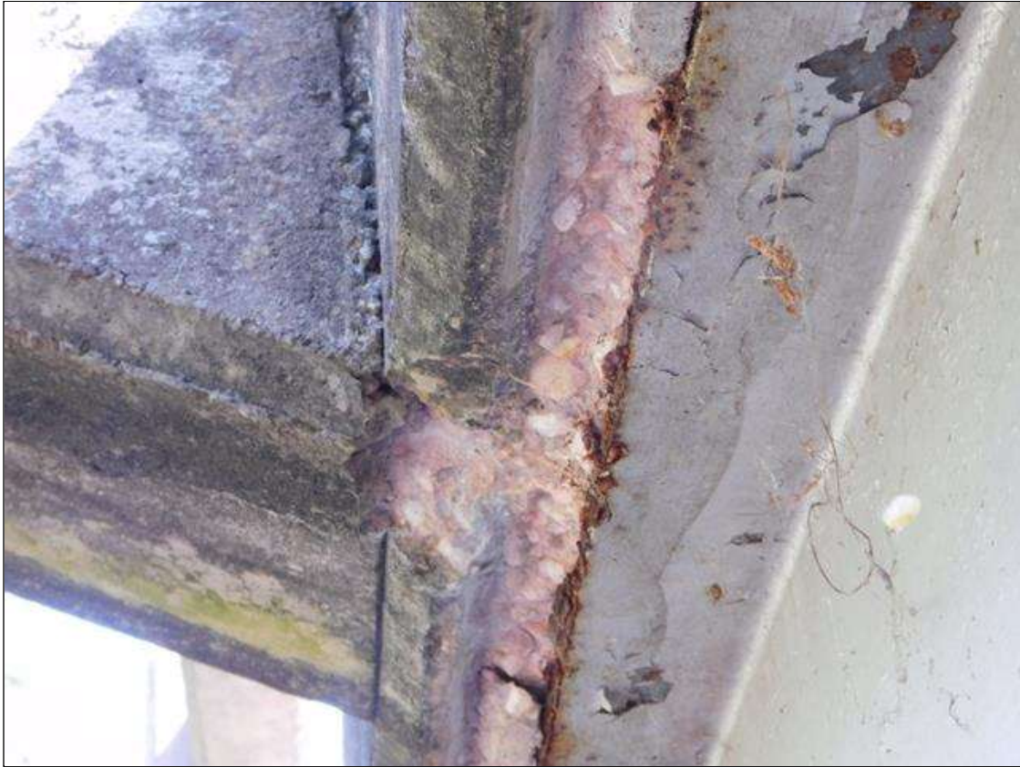
Span 2 Deck: 18" x 3" x 1" DEEP SPALL IN LEFT OVERHANG. LOCATED 4' FROM END BENT 2.
