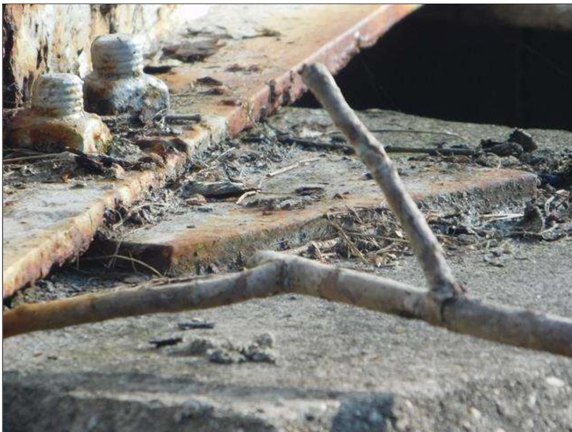
Span 1 Beam 11 - Span 1 Beam 11 Far Bearing: SURFACE RUST, BEARING ASSEMBLY.
