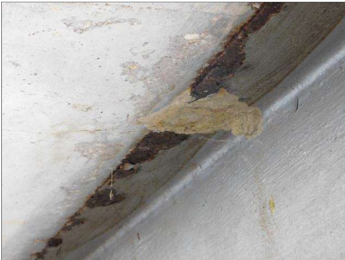
Span 2 Beam 10: 5' OF RUST SCALE, TOP FLANGE, NEAR MID-SPAN.
