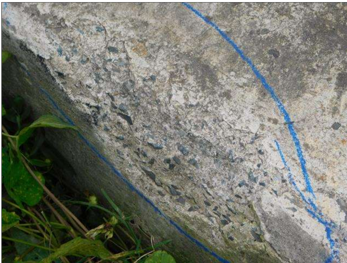
Span 1 Right Bridge Rail: top of curb at End Bent 1, spall [8in x 6in x 3/4in]
