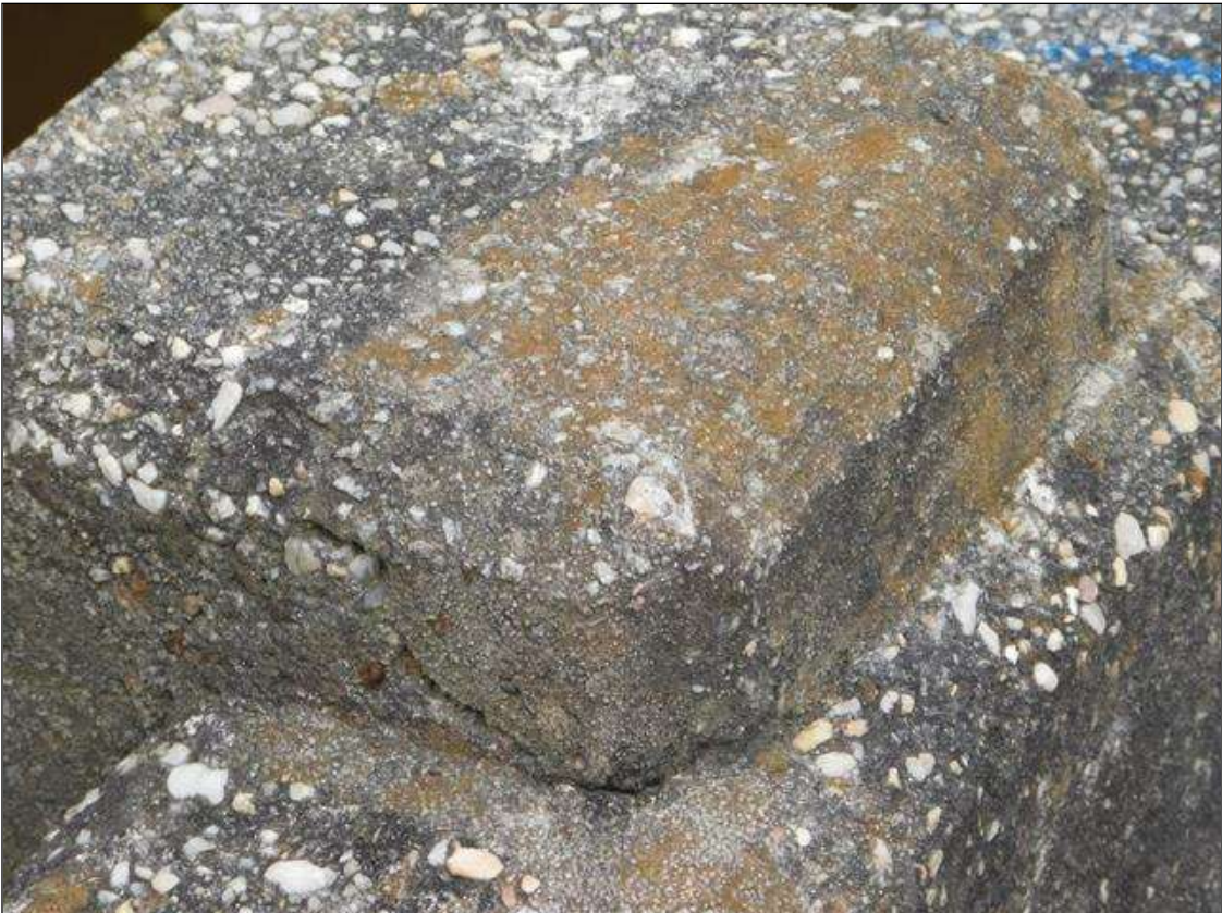
Span 1 Left Bridge Rail: at top of rail post 2 and 3, delamination [7in x 3in]
