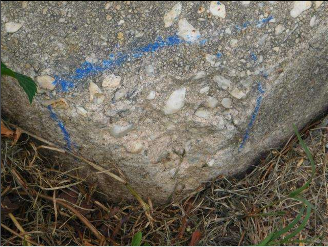
Span 1 Left Bridge Rail: 4" X UP TO 4" X 1/2" SPALL, SOUTHEAST CORNER OF BOTTOM RAIL, AT END BENT 1.
