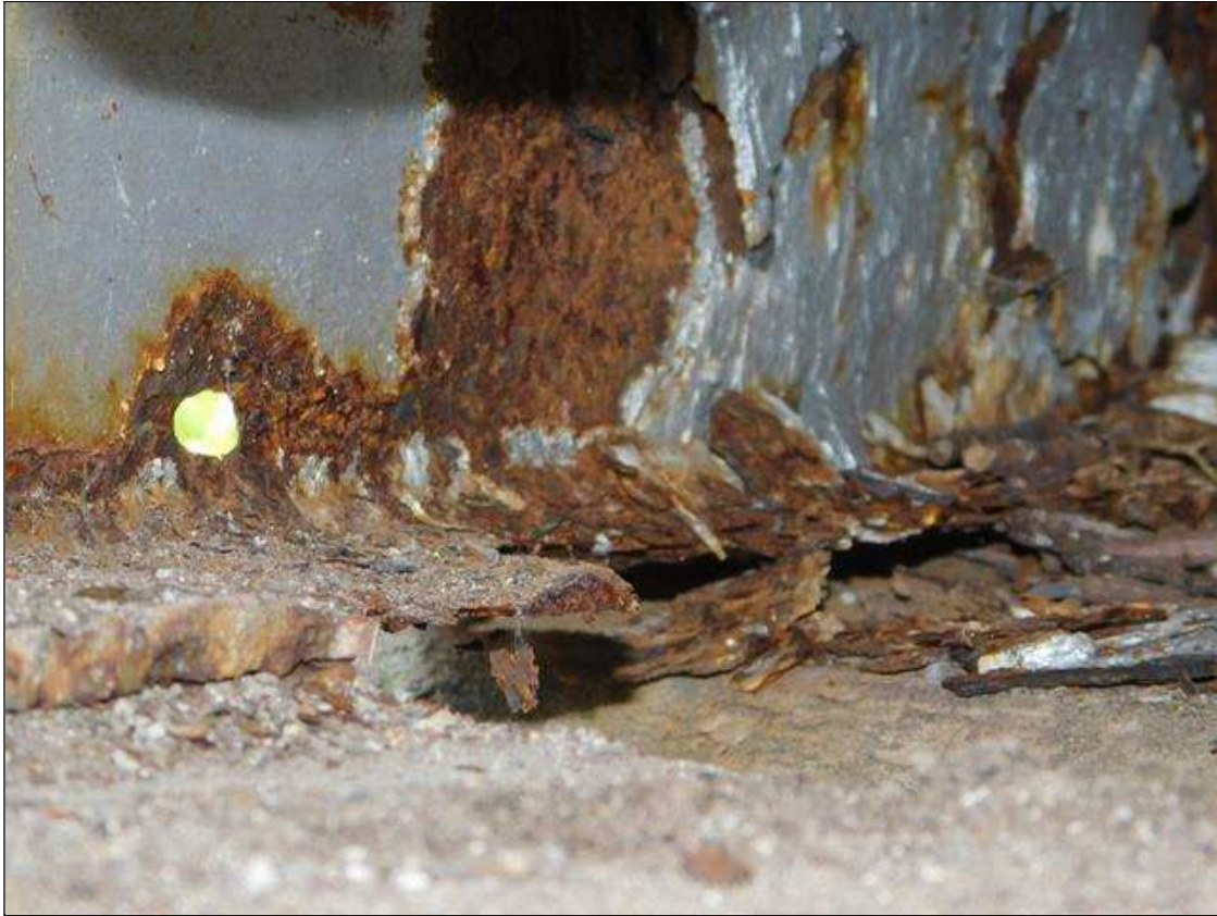
Span 2 Beam 11: 3' OF RUST SCALE IN TOP FLANGE WITH 5/16" REMAINING. BOTTOM FLANGE HAS A 12" x 3" AREA OF 100% SECTION LOSS. WEB HAS A 1 1/2" DIAMETER HOLE. THESE AREAS ARE OVER BENT 1. A "PAR" HAS BEEN ISSUED FOR THESE CONDITIONS.
