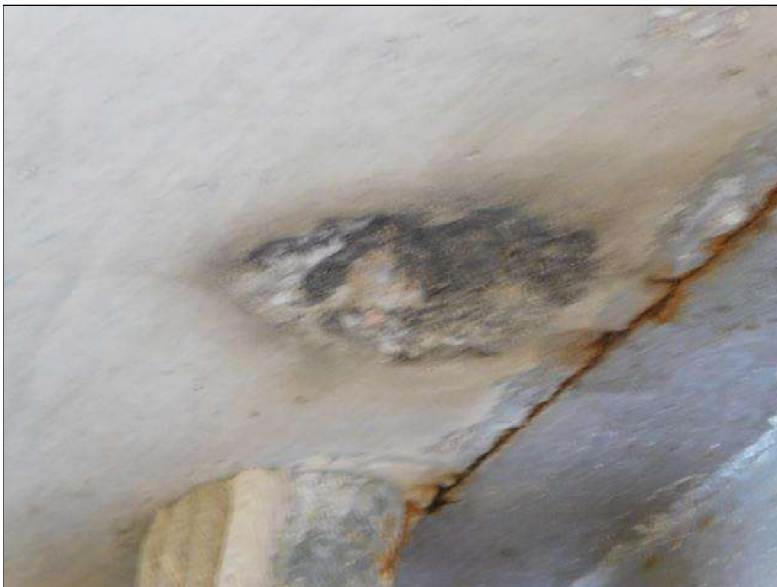
Span 2 Deck: 3" DIAMETER X 1" SPALL, WITH EXPOSED REINFORCING, DECK UNDERSIDE, BAY 1, 2' FROM BENT 1.
