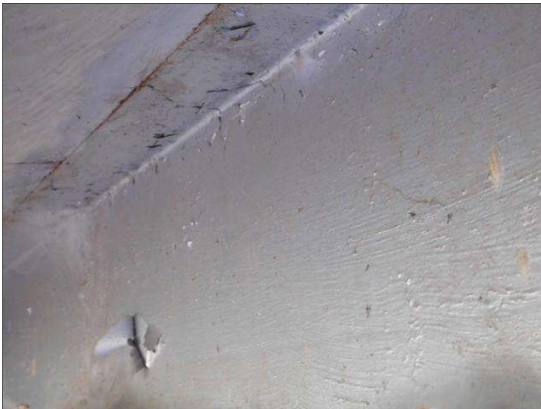
Span 2 Beam 3 - Protective System: along length of beam, bubbling paint in surface coat only
