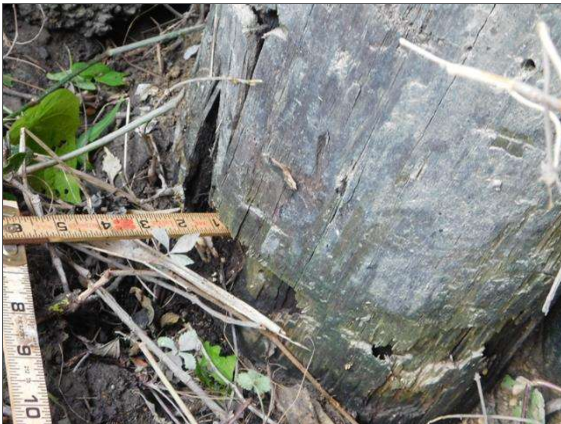
End Bent 1 Pile 5: END BENT 1 PILE 5 NORTH FACE. HAS A 12" x 10" x 1" DEEP AREA OF HEAVY DECAY AT GROUND LINE.
