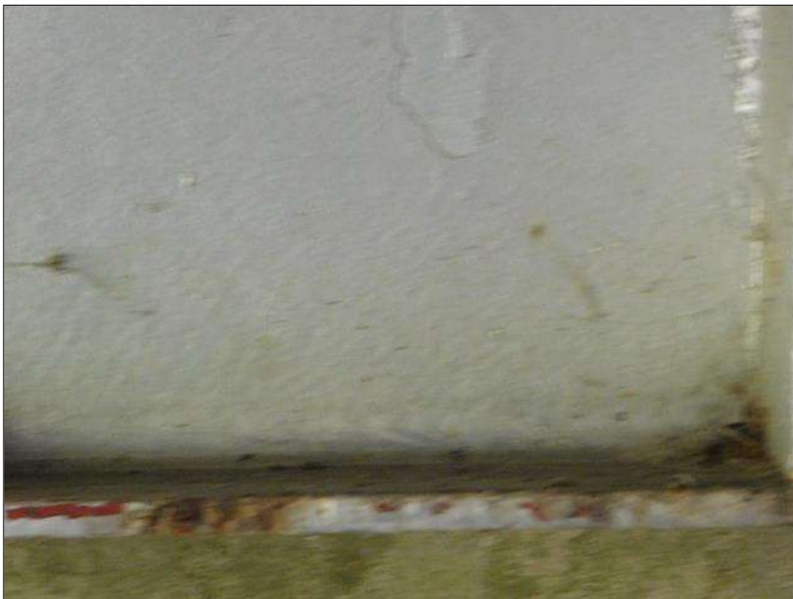
Span 1 Crutch Bent 1 Cap 1: along length of cap, random areas of surface corrosion with no section loss
