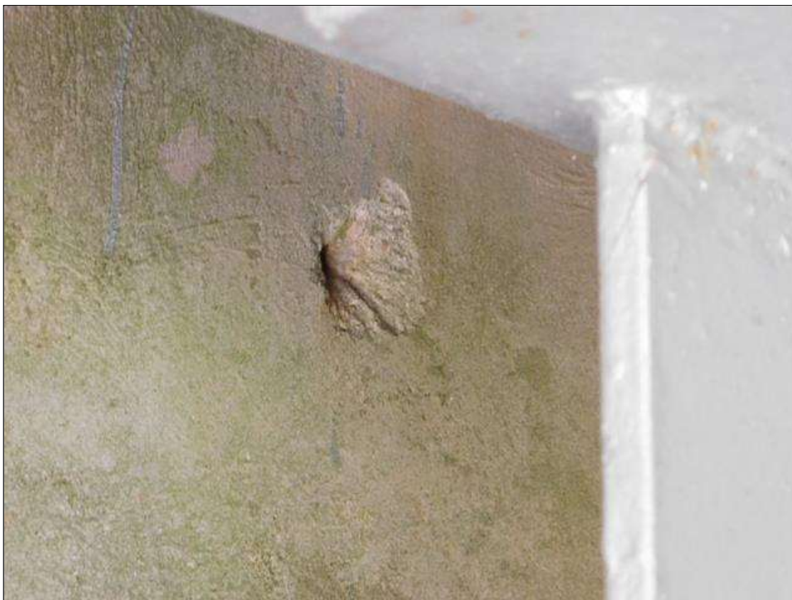
Bent 1 Cap 1: 2" DIAMETER X 3/4" SPALL, WITH EXPOSED REINFORCING, NORTH FACE OF CAP, 3' EAST OF PILE 3.
