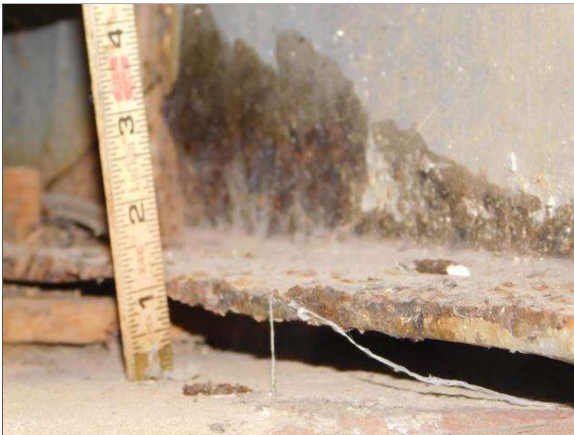
Span 2 Beam 9: 1' OF RUST SCALE, BOTTOM FLANGE, UP TO 2" IN THE WEB, WITH 1/8" REMAINING IN THE BOTTOM FLANGE, AT BENT 1. A "PAR" HAS BEEN ISSUED FOR THIS CONDITION.
