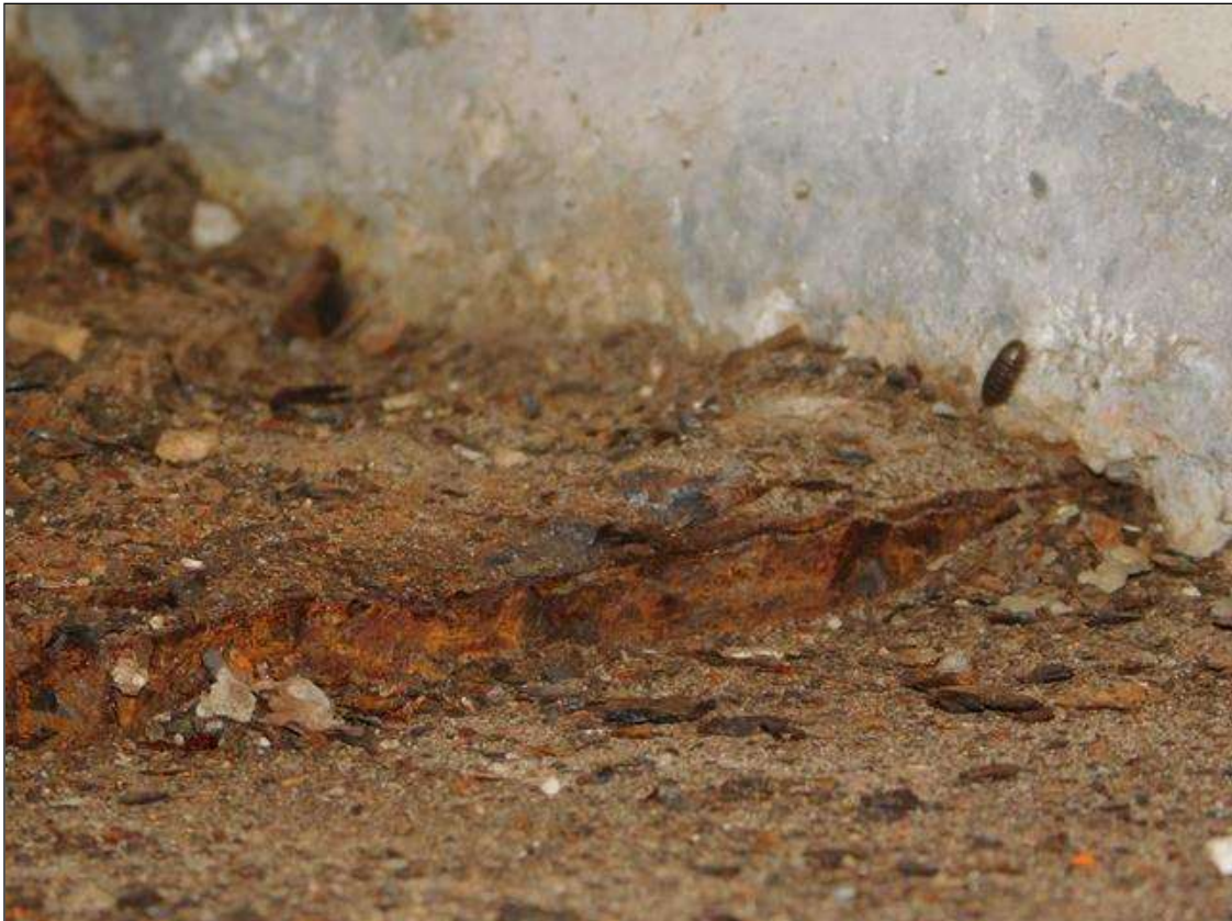
Span 2 Beam 1 - Span 2 Beam 1 Far Bearing: surface corrosion with no section loss noted
