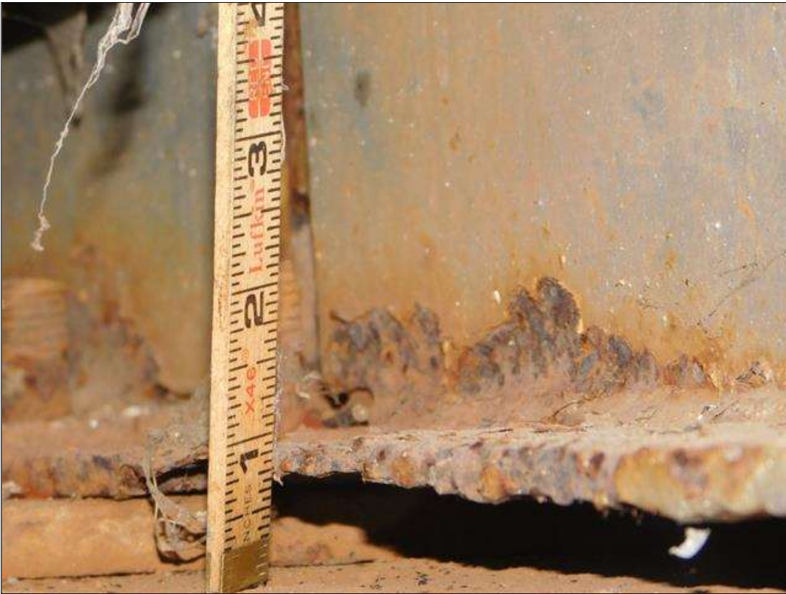
Span 1 Beam 4: 6" OF RUST SCALE, BOTTOM FLANGE, UP TO 3" IN THE WEB DOWN TO A KNIFE EDGE REMAINING IN THE BOTTOM FLANGE, AT BENT 1. A "PAR" HAS BEEN ISSUED FOR THIS CONDITION.
