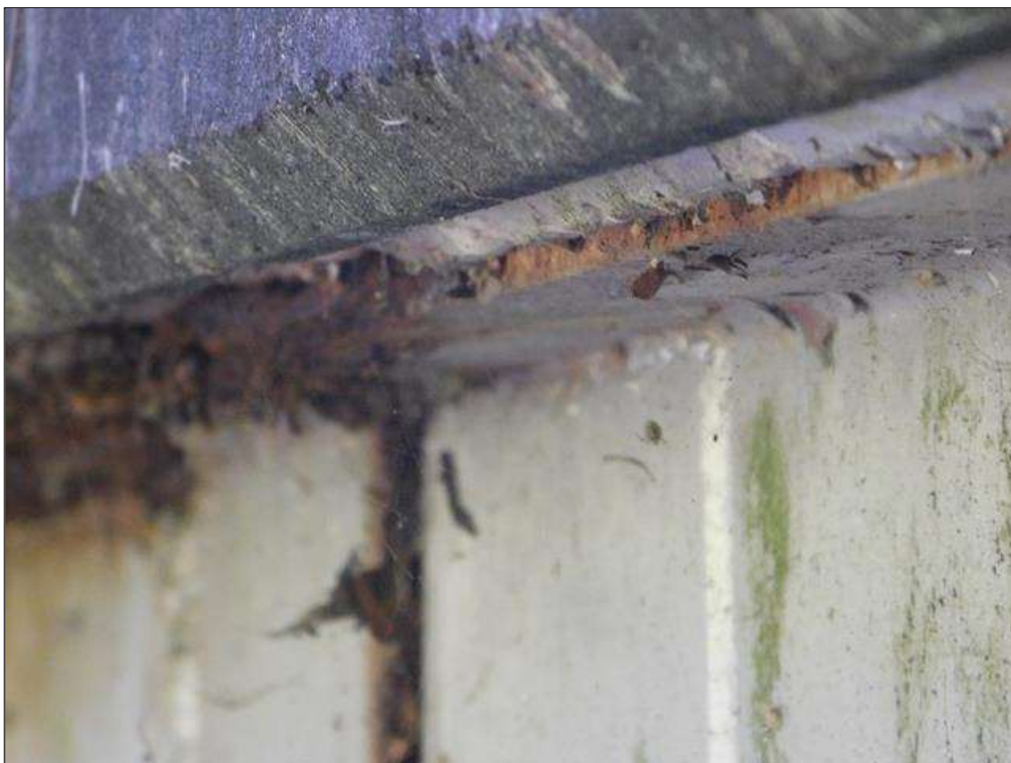
Span 1 Beam 1: at near and far ends, surface corrosion [up to full height x full width]
