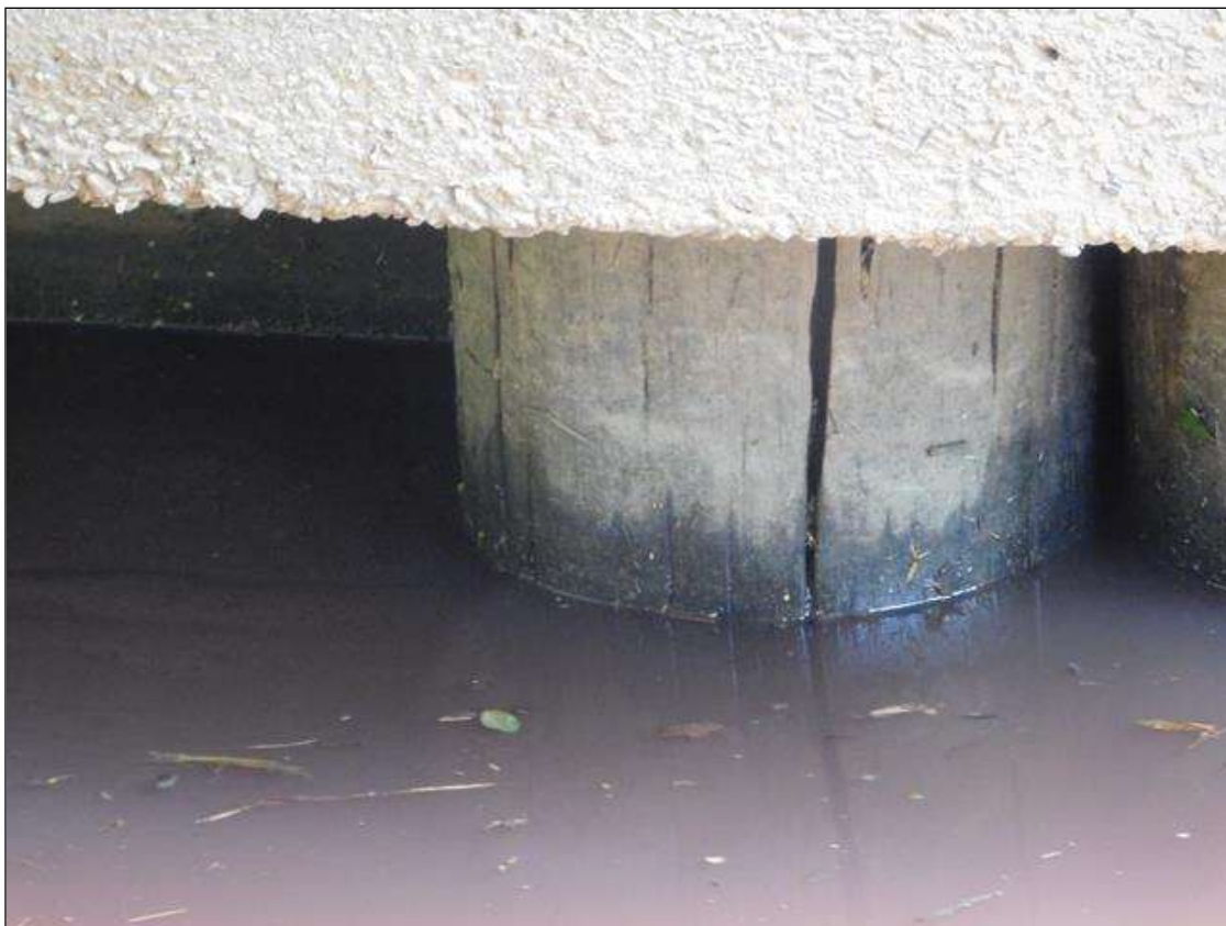
End Bent 2 Pile 5: at exposed pile below concrete collar, checks [3/8in x 3/4in deep]
