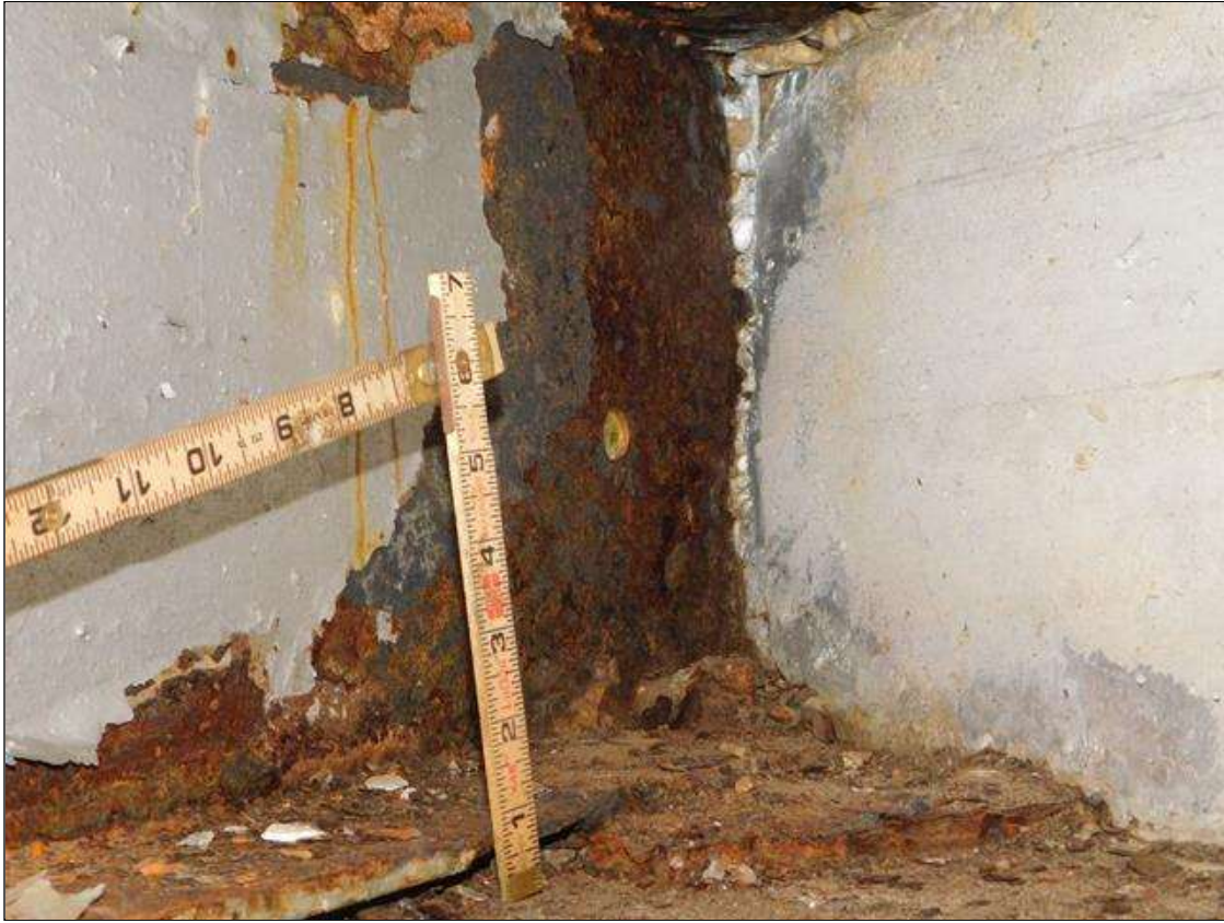
Span 2 Beam 1: SPAN 2 BEAM 1 OVER END BENT 1. WEB AND FLANGES HAVE AREAS OF SECTION LOSS WITH 1/8" REMAINING IN BOTTOM FLANGE AND 3/16" REMAINING IN WEB. AREA IS: FROM END OF BEAM OUT 18" x FULL WIDTH OF FLANGE AND FROM END OF BEAM OUT 12" x FULL HEIGHT OF WEB. A "PAR" HAS BEEN ISSUED FOR THESE CONDITIONS.
