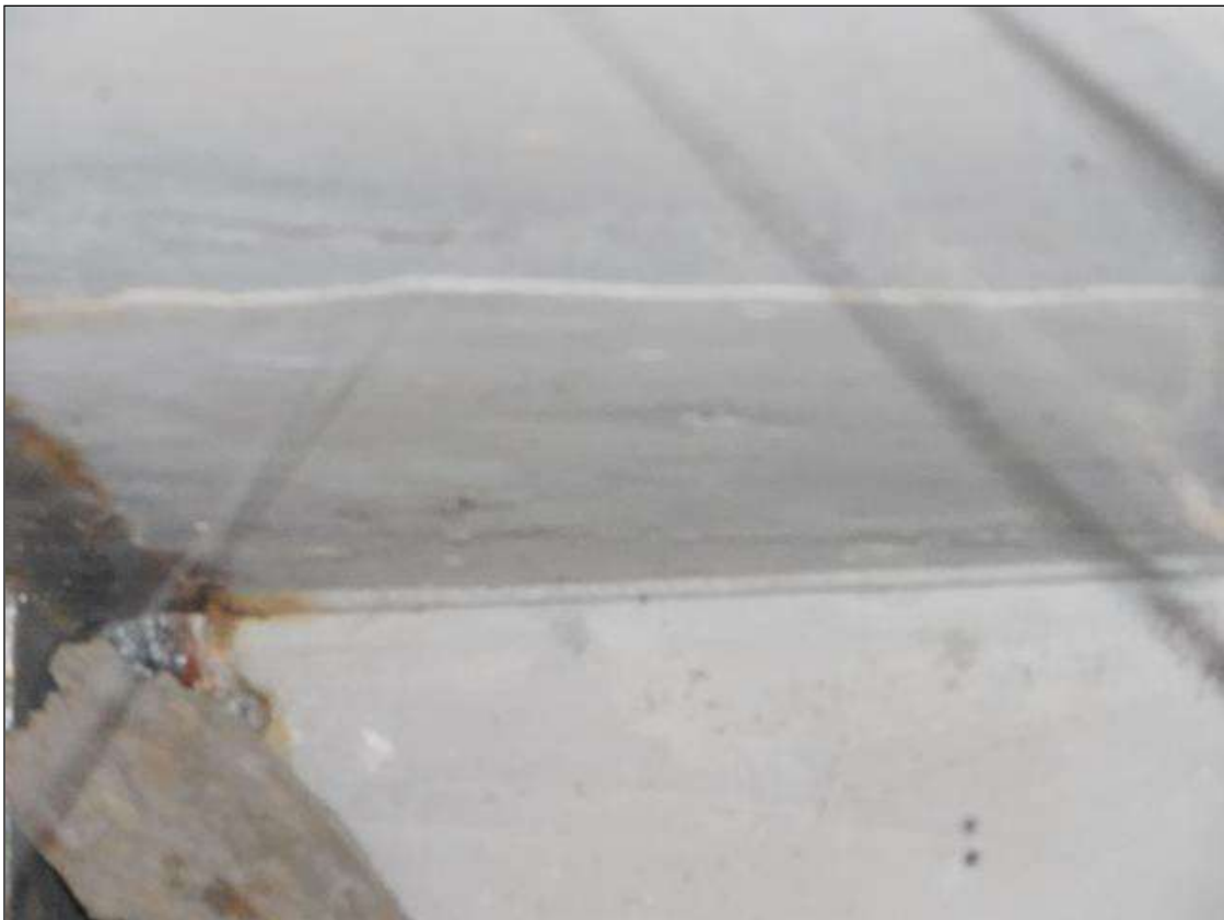
Span 1 Deck: 2.5' X 2' PATCHED AREA, DECK UNDERSIDE, BAY 4, AT BENT 1.
