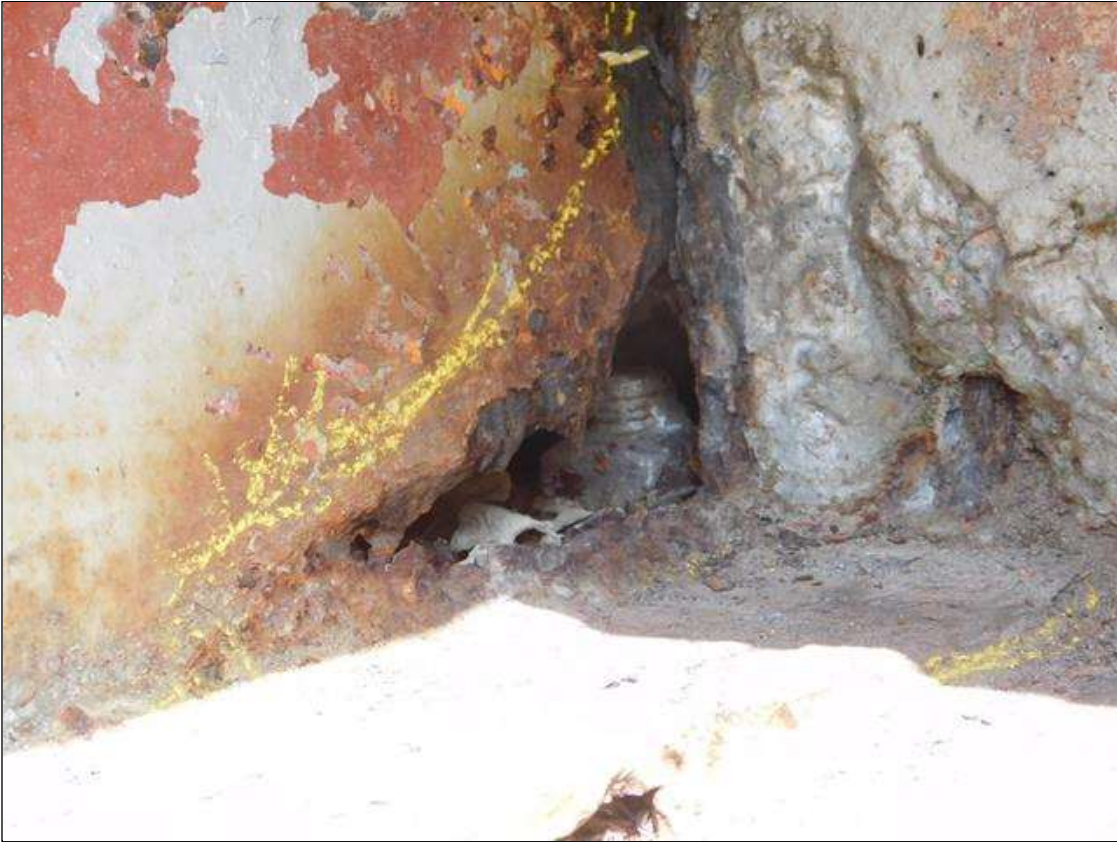
Span 2 Beam 11: SPAN 2 BEAM 11 RIGHT WEB AND BOTTOM FLANGE OVER END BENT 2. WEB HAS A 5" x 3" AREA OF 100% SECTION LOSS. BOTTOM FLANGE HAS A 7" x 3" AREA OF SECTION LOSS WITH 1/4" REMAINING. A "PAR" HAS BEEN ISSUED FOR THIS CONDITION.
