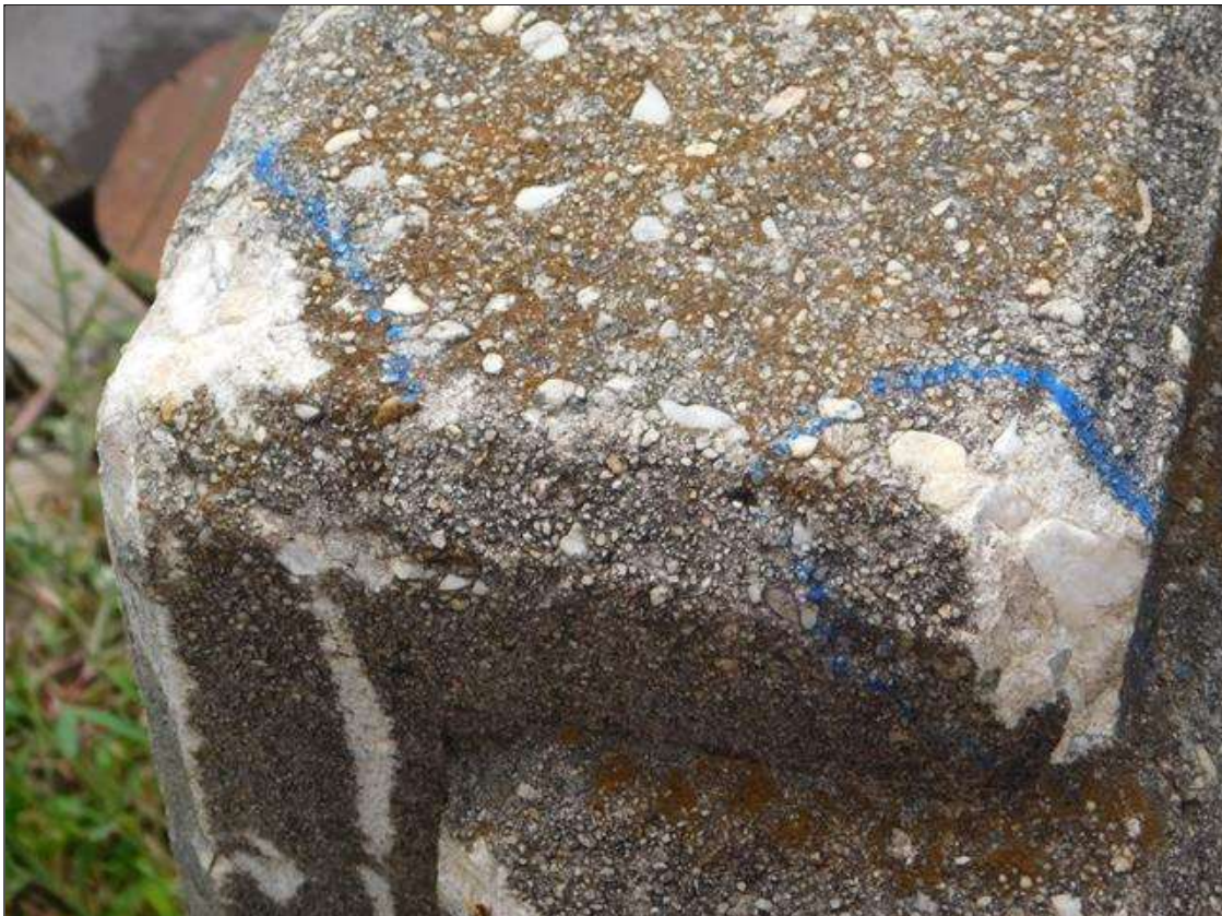
Span 2 Right Bridge Rail: RIGHT RAIL TOP OF END POST AT NORTH END. HAS (2) SPALLED AREAS. AREAS ARE: 2" x 1" x 1/4" DEEP AND 3" x 2" x 1/4" DEEP.
