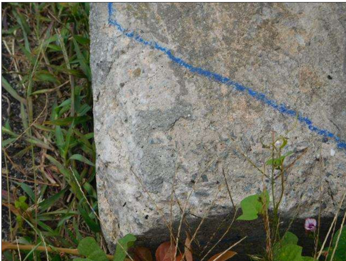
Span 2 Left Bridge Rail: LEFT RAIL NORTHEAST CORNER OF CURB. HAS A 10" x 8" x 1/2" DEEP SPALL.
