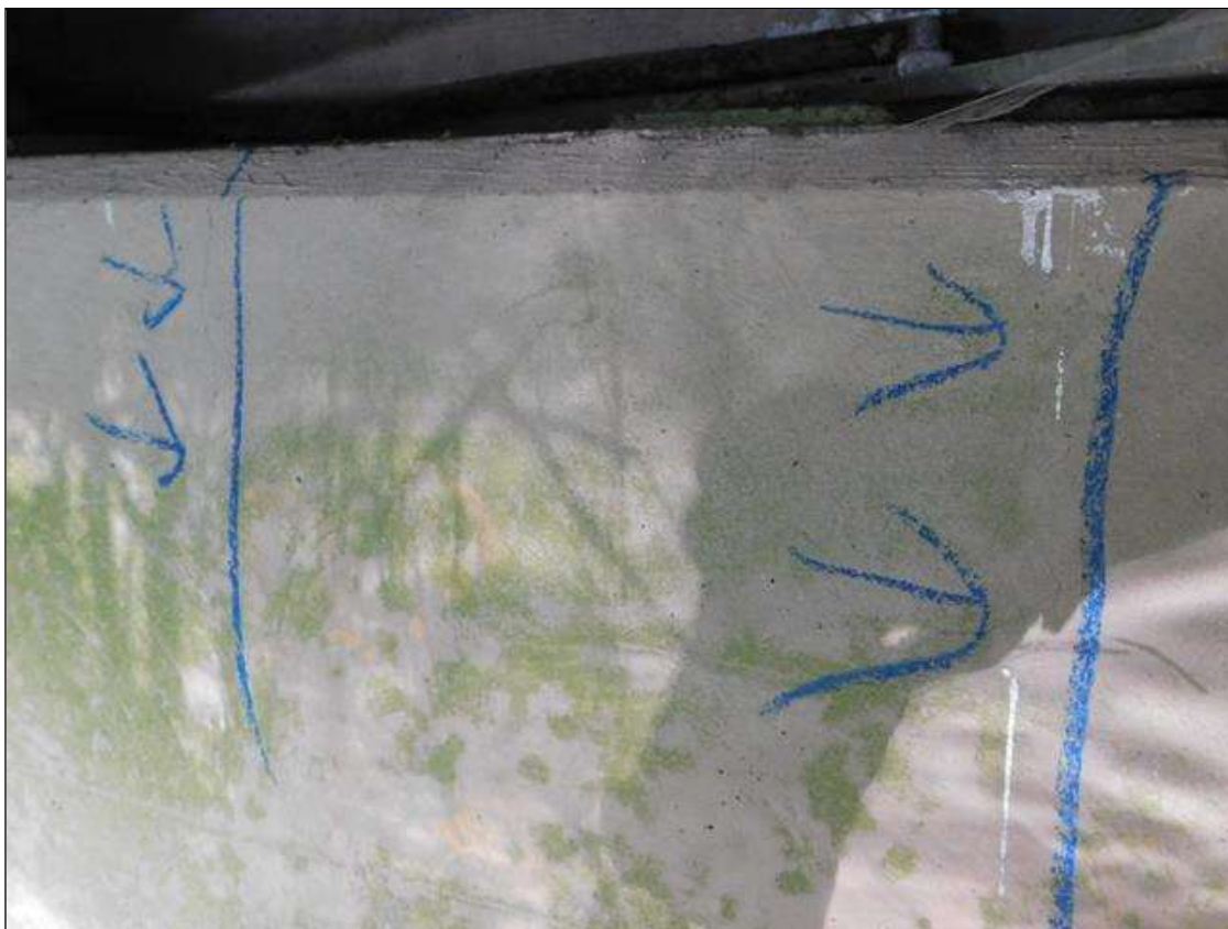
End Bent 1 Cap 1: at bay 9, (2) vertical cracks [1ft x 0.02in]
