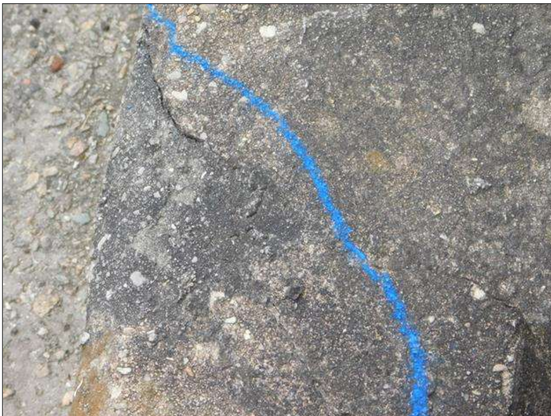
Span 2 Left Bridge Rail: top face of curb at bent 1, diagonal crack [14in x 0.02in]
