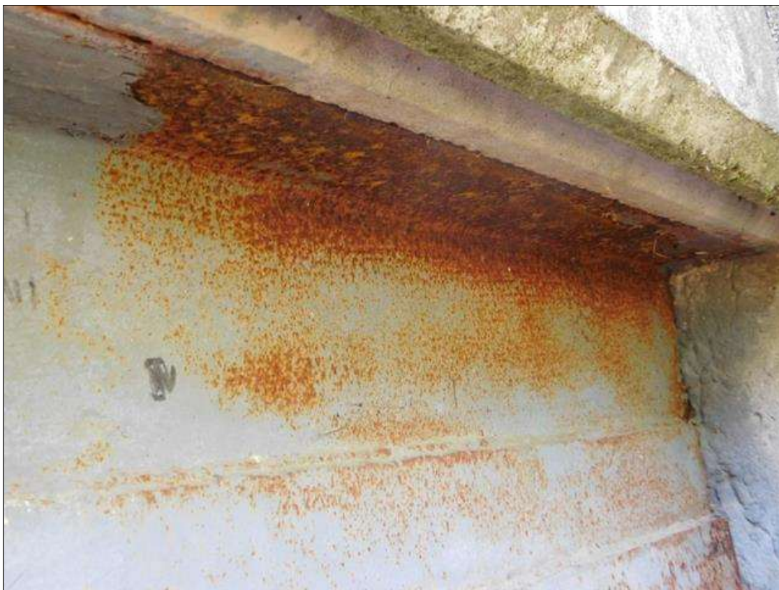
Span 1 Beam 1: 2' OF FRECKLED RUST, TOP AND BOTTOM FLANGE AND WEB, WEST FACE, AT END BENT 1.
