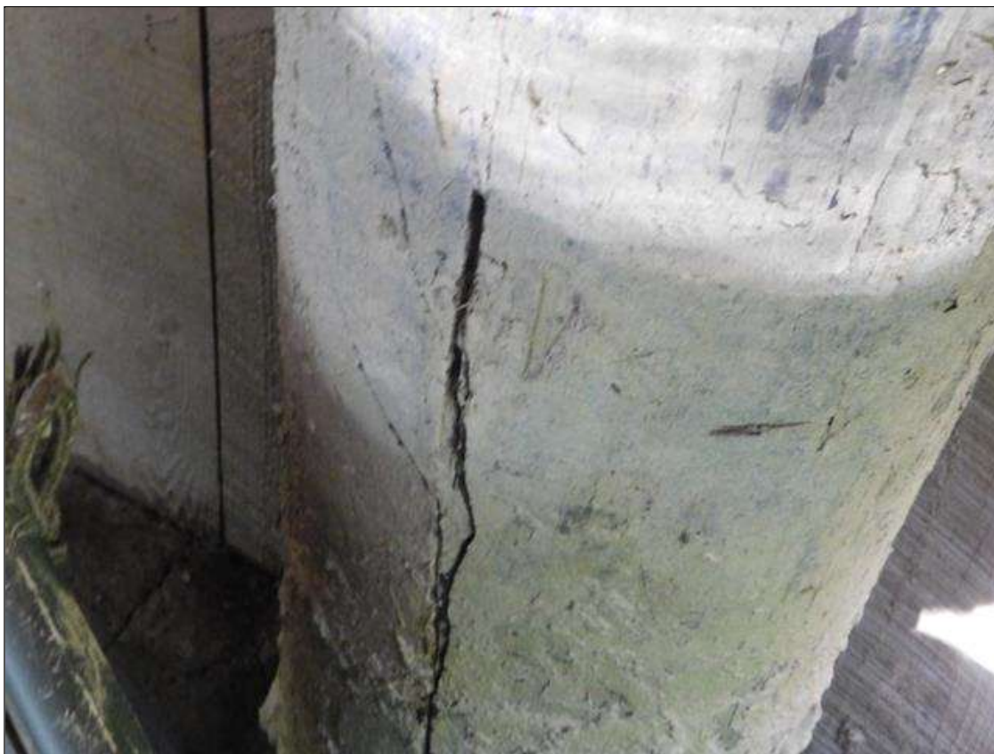
End Bent 1 Pile 2: UP TO 2' X 1/8" X 1/2" CHECKS, AT RANDOM THROUGHOUT.
