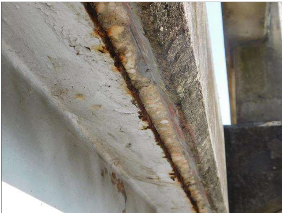
Span 1 Deck: 21' X 2" X 1" SPALL, DECK UNDERSIDE, RIGHT OVERHANG, AT BENT 1.
