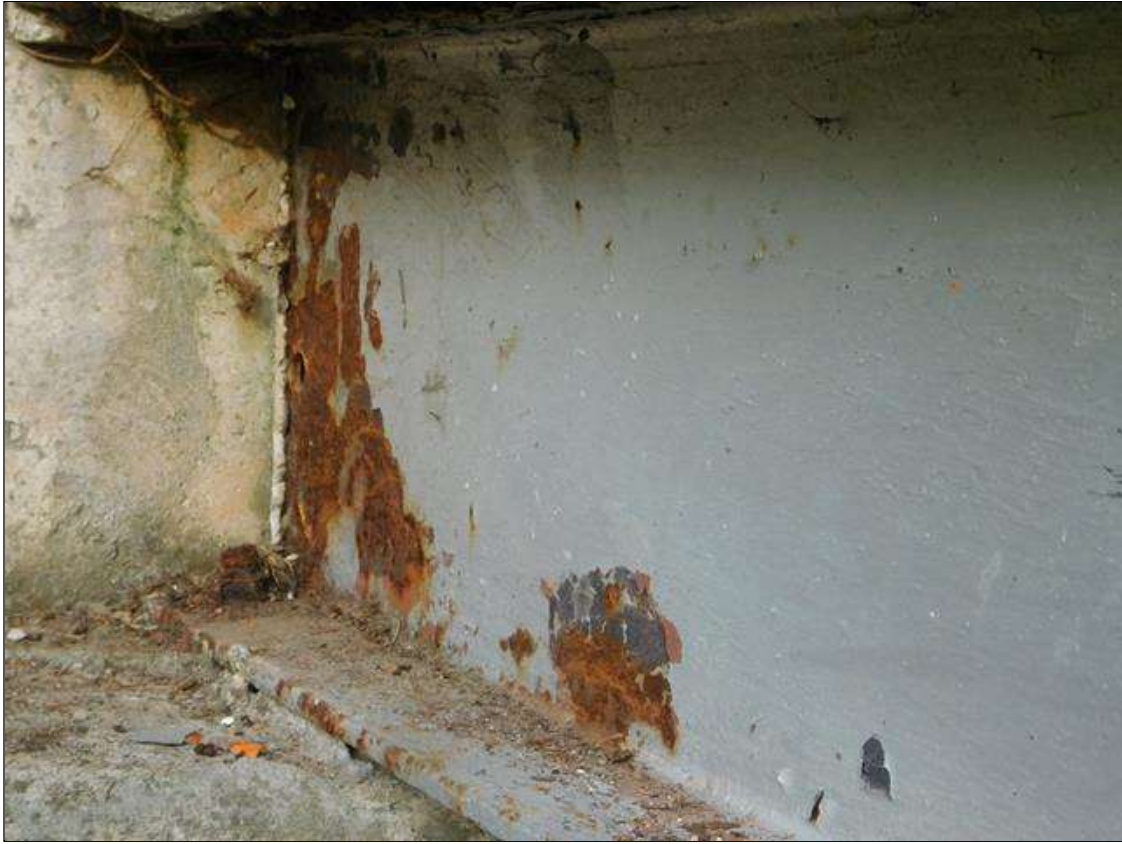
Span 1 Beam 11: at near and far ends, surface corrosion [up to full height x full width]
