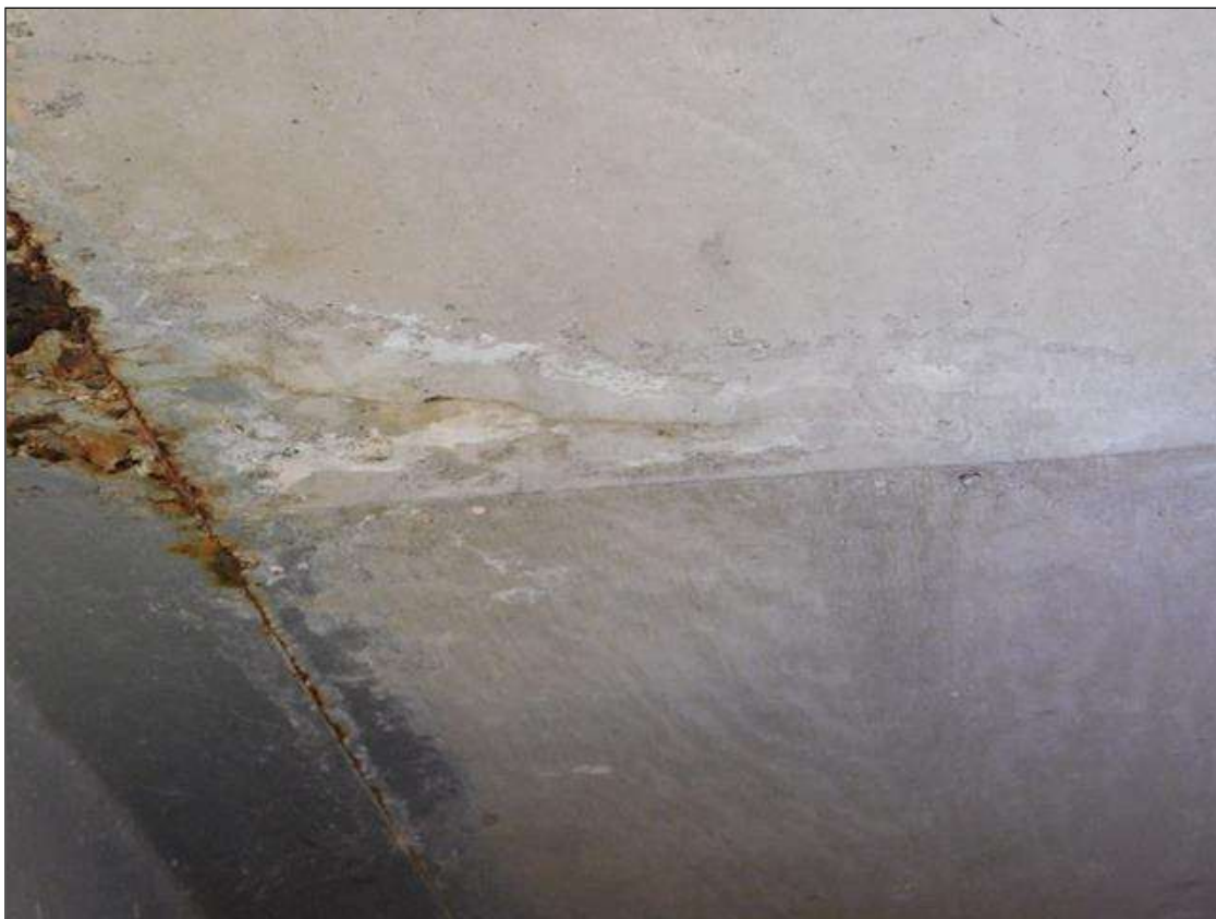
Span 2 Deck: 2' X 1/16" CRACK, WITH EFFLORESCENCE, DECK UNDERSIDE, BAY 2, AT END BENT 2.
