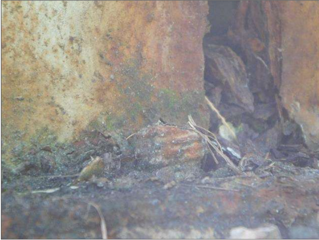
Span 2 Beam 1: West side at near end, anchor bolt nut is missing
