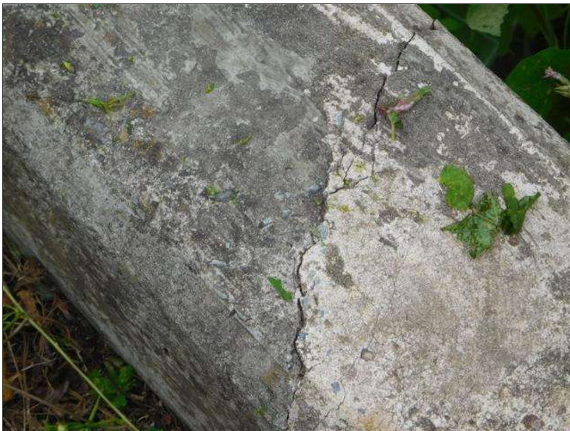
Span 1 Right Bridge Rail: top face of curb at End Bent 1, diagonal crack [8in x 0.02in]
