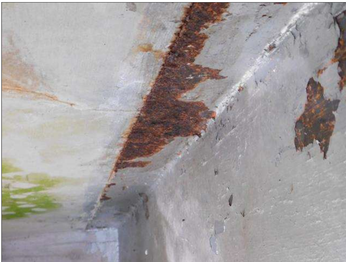
Span 1 Beam 10: BEAM 10 TOP FLANGE. HAS SCATTERED AREAS OF RUST AND FLAKING WITH NO MEASURABLE SECTION LOSS.
