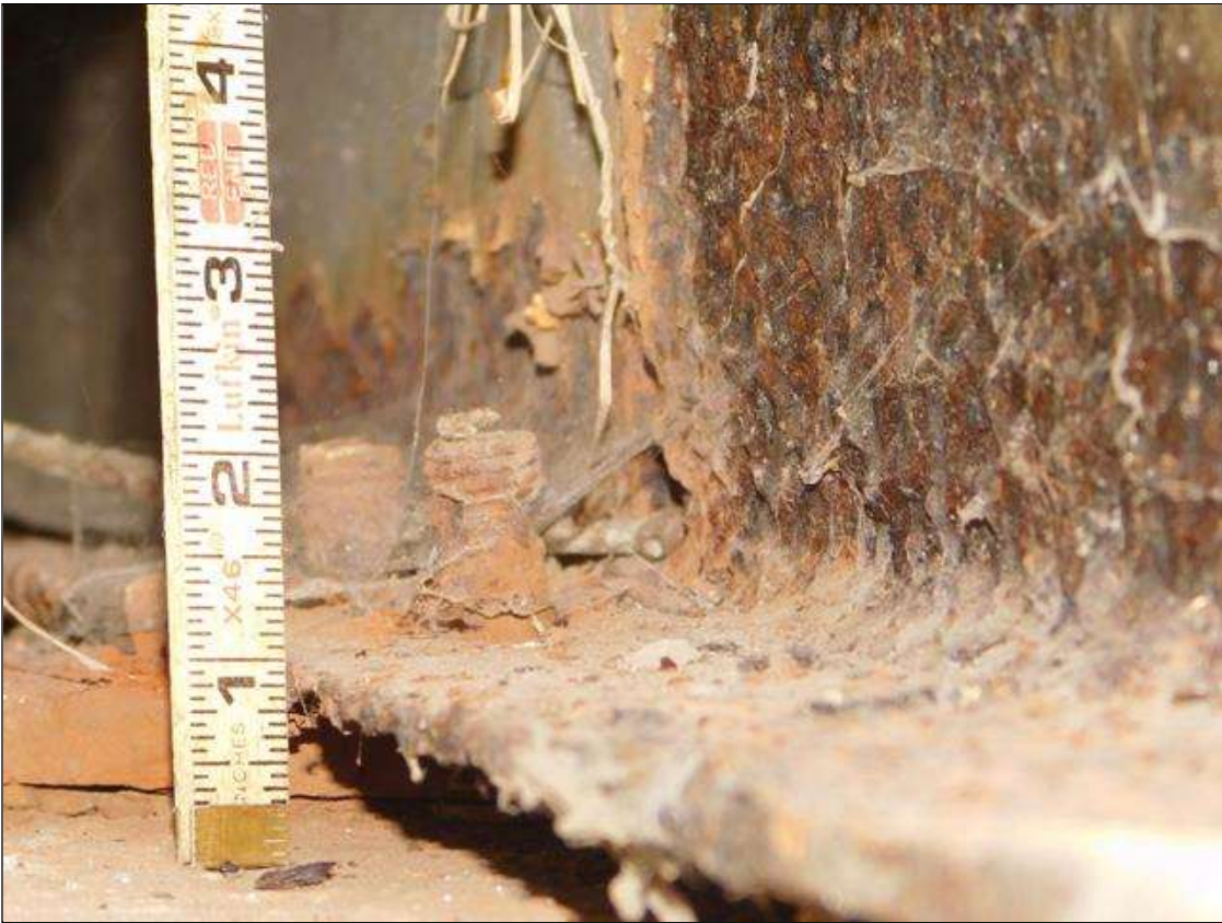
Span 1 Beam 6: 1' OF RUST SCALE, BOTTOM FLANGE, UP TO 5" IN THE WEB, WITH 1/8" REMAINING IN THE BOTTOM FLANGE, AT BENT 1. A "PAR" HAS BEEN ISSUED FOR THIS CONDITION.
