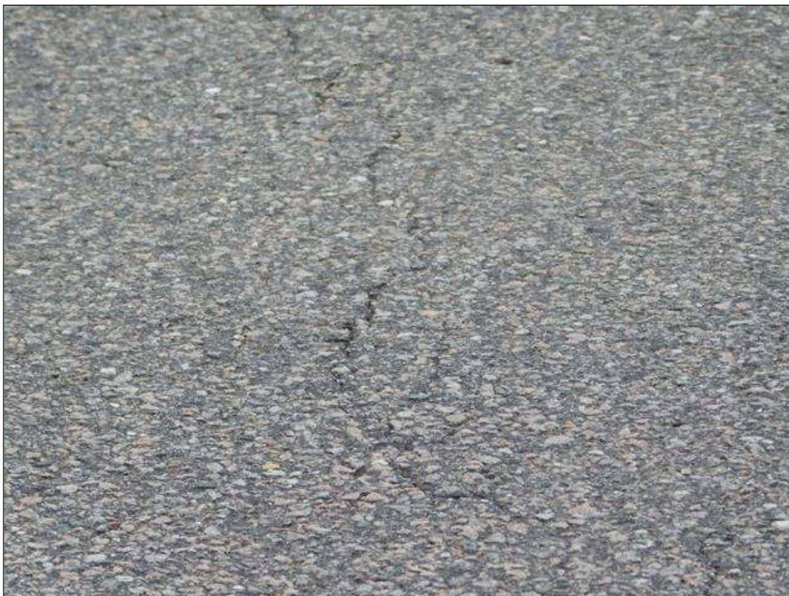
Span 1 Wearing Surface: throughout span, multiple transverse cracks [full width x up to 0.02in]
