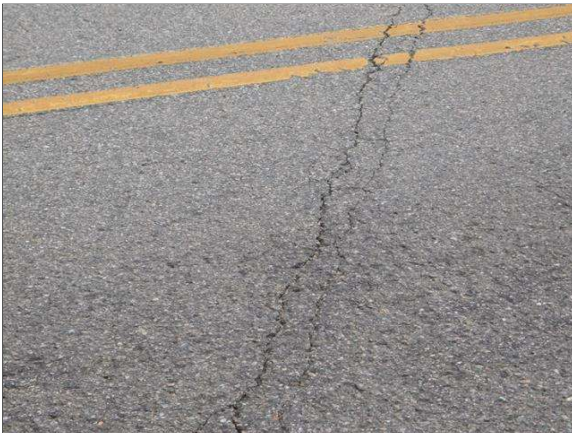
Span 2 Wearing Surface: at bent 1 and End Bent 2, transverse crack [full width x 1/8in]
