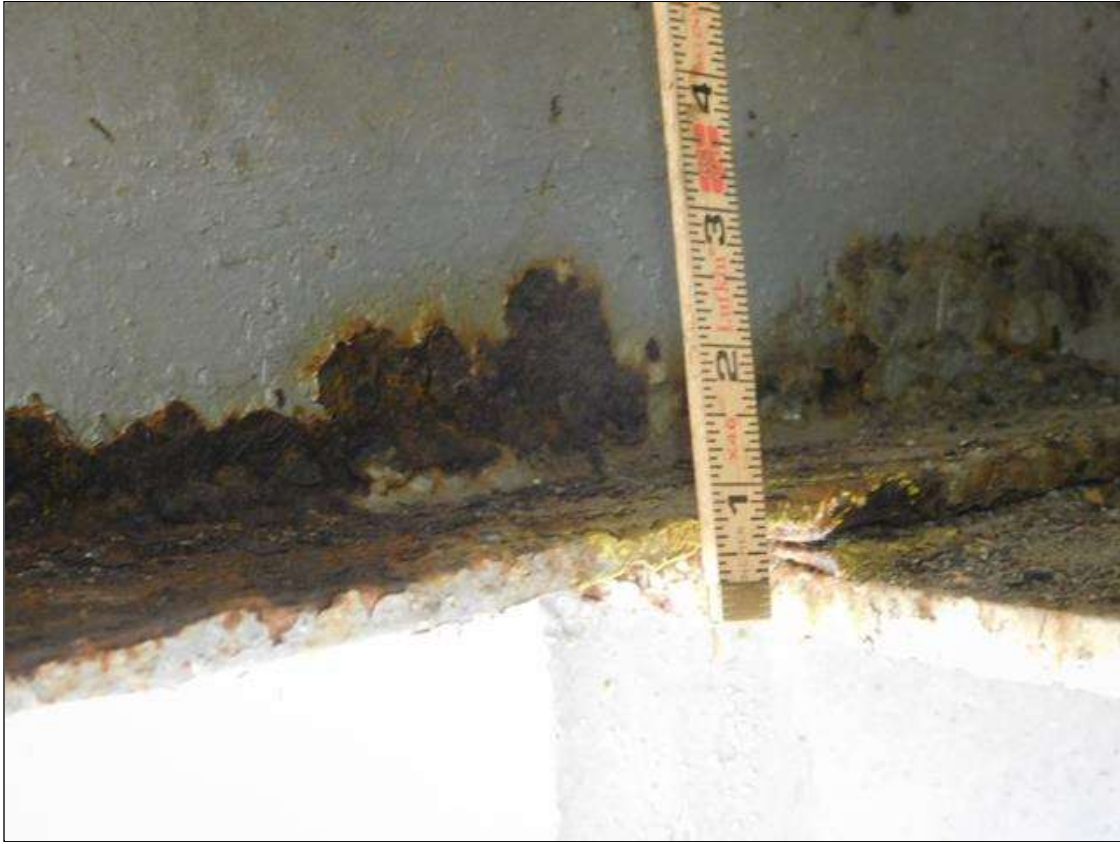
Span 2 Beam 11: BEAM 11 LEFT BOTTOM FLANGE AT CRUTCH BENT. HAS A AREA OF SECTION LOSS WITH 1/4" REMAINING. AREA IS: 3" WIDE x 10" LONG. A "PAR" HAS BEEN ISSUED FOR THIS CONDITION.
