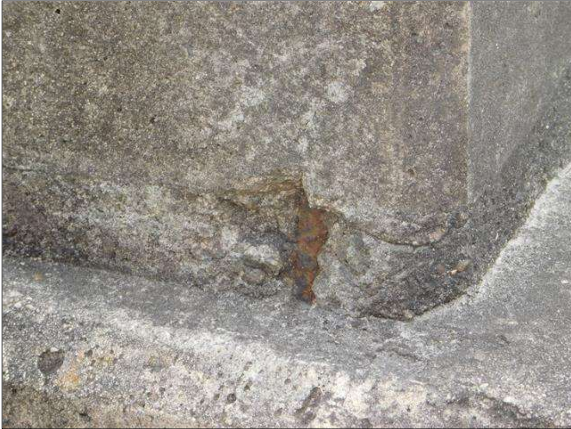
Span 2 Right Bridge Rail: at base of rail post 1, spall [2in x 2in x 1/2in deep] with exposed rusted reinforcing no section loss noted
