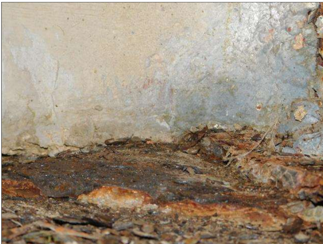
Span 1 Beam 1 - Span 1 Beam 1 Near Bearing: surface corrosion with section loss [1/16in]
