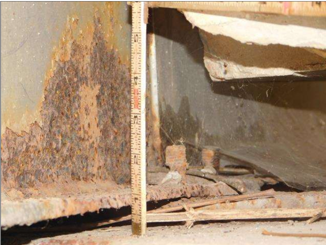
Span 1 Beam 7: 18" OF RUST SCALE, BOTTOM FLANGE, UP TO 5" IN THE WEB, 1/4" REMAINING IN THE BOTTOM FLANGE, AT BENT 1. A "PAR" HAS BEEN ISSUED FOR THIS CONDITION.
