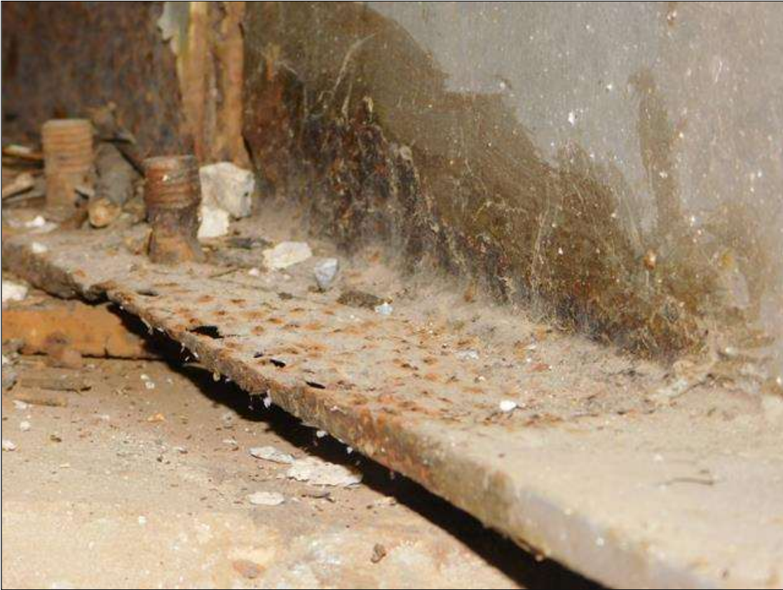
Span 2 Beam 8: 1' OF RUST SCALE, BOTTOM FLANGE, UP TO 2" IN THE WEB, WITH 1/16" REMAINING IN THE BOTTOM FLANGE, AT BENT 1. BOTTOM FLANGE HAS (3) 1" DIAMETER HOLES. A "PAR" HAS BEEN ISSUED FOR THIS CONDITION.
