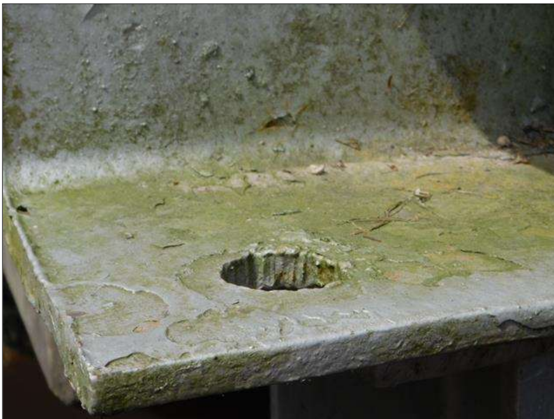
Span 2 Crutch Bent 2 Cap 1: 1" DIAMETER HOLE, BOTTOM FLANGE, EAST END OF CAP.
