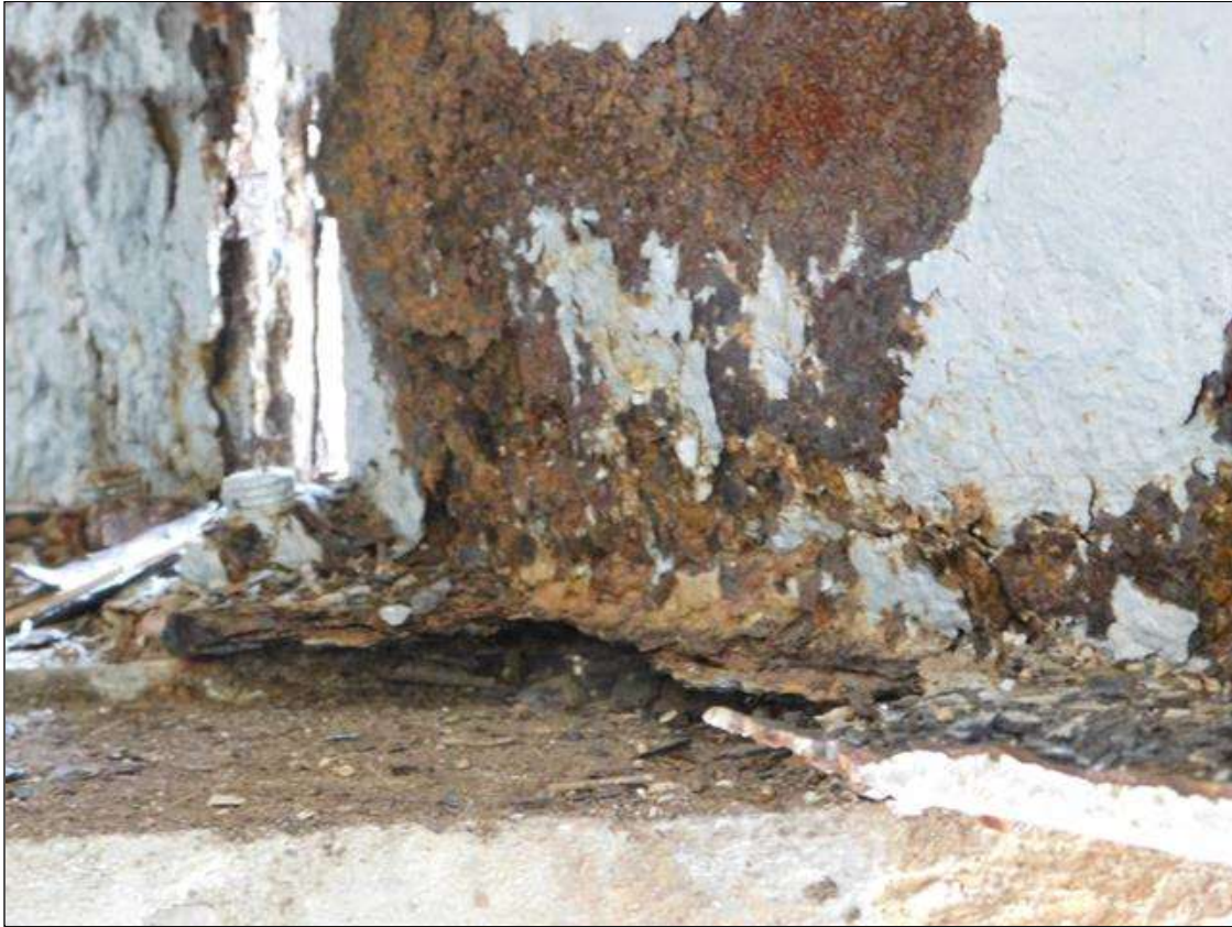
Span 1 Beam 11: 3' OF RUST SCALE, TOP AND BOTTOM FLANGE, UP TO 6" IN THE WEB, WITH 6" X UP TO 3" HOLE IN THE BOTTOM FLANGE, WITH 3/8" REMAINING IN THE WEB, WITH 5/16" REMAINING IN THE BOTTOM FLANGE, AT BENT 1. A "PAR" HAS BEEN ISSUED FOR THIS CONDITION.
