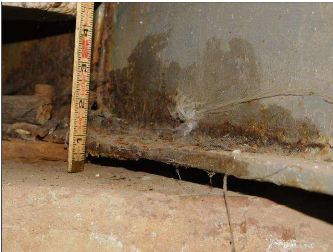
Span 2 Beam 5: 1' OF RUST SCALE, BOTTOM FLANGE, UP TO 2" IN THE WEB, WITH 1/4" REMAINING IN THE BOTTOM FLANGE, AT BENT 1. A "PAR" HAS BEEN ISSUED FOR THIS CONDITION.
