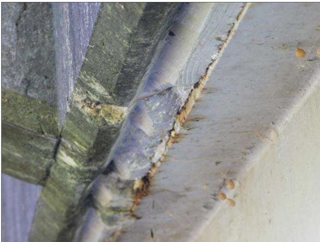
Span 1 Deck: 1' X 2" X 1" SPALL, DECK UNDERSIDE, LEFT OVERHANG, AT BENT 1.
