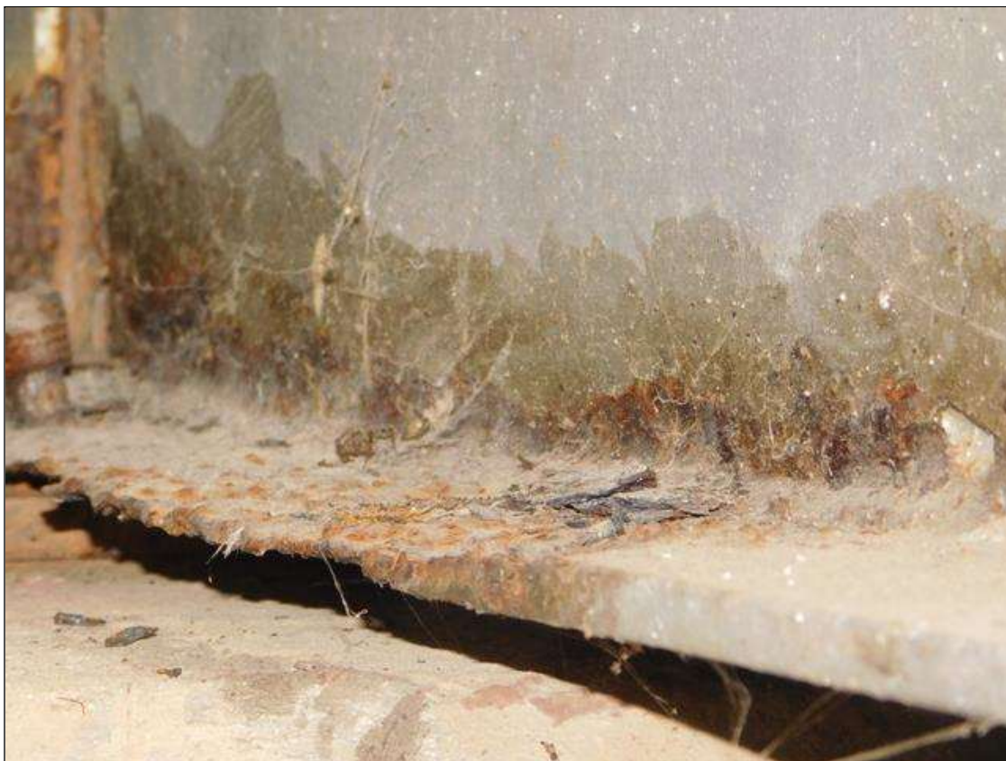
Span 2 Beam 7: 1' OF RUST SCALE, BOTTOM FLANGE, UP TO 2" IN THE WEB, WITH A KNIFE EDGE REMAINING IN THE BOTTOM FLANGE, AT BENT 1. A "PAR" HAS BEEN ISSUED FOR THIS CONDITION.
