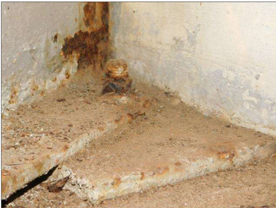
Span 1 Beam 11 - Span 1 Beam 11 Near Bearing: surface corrosion in bearing plate with a 1/16" section loss anchor bolt nut on left and right side.
