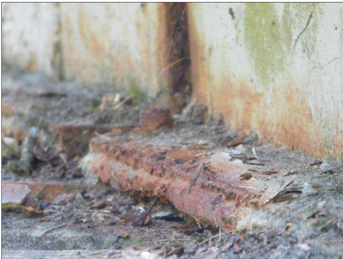
Span 1 Beam 1 - Span 1 Beam 1 Far Bearing: at West side anchor bolt nut is missing
