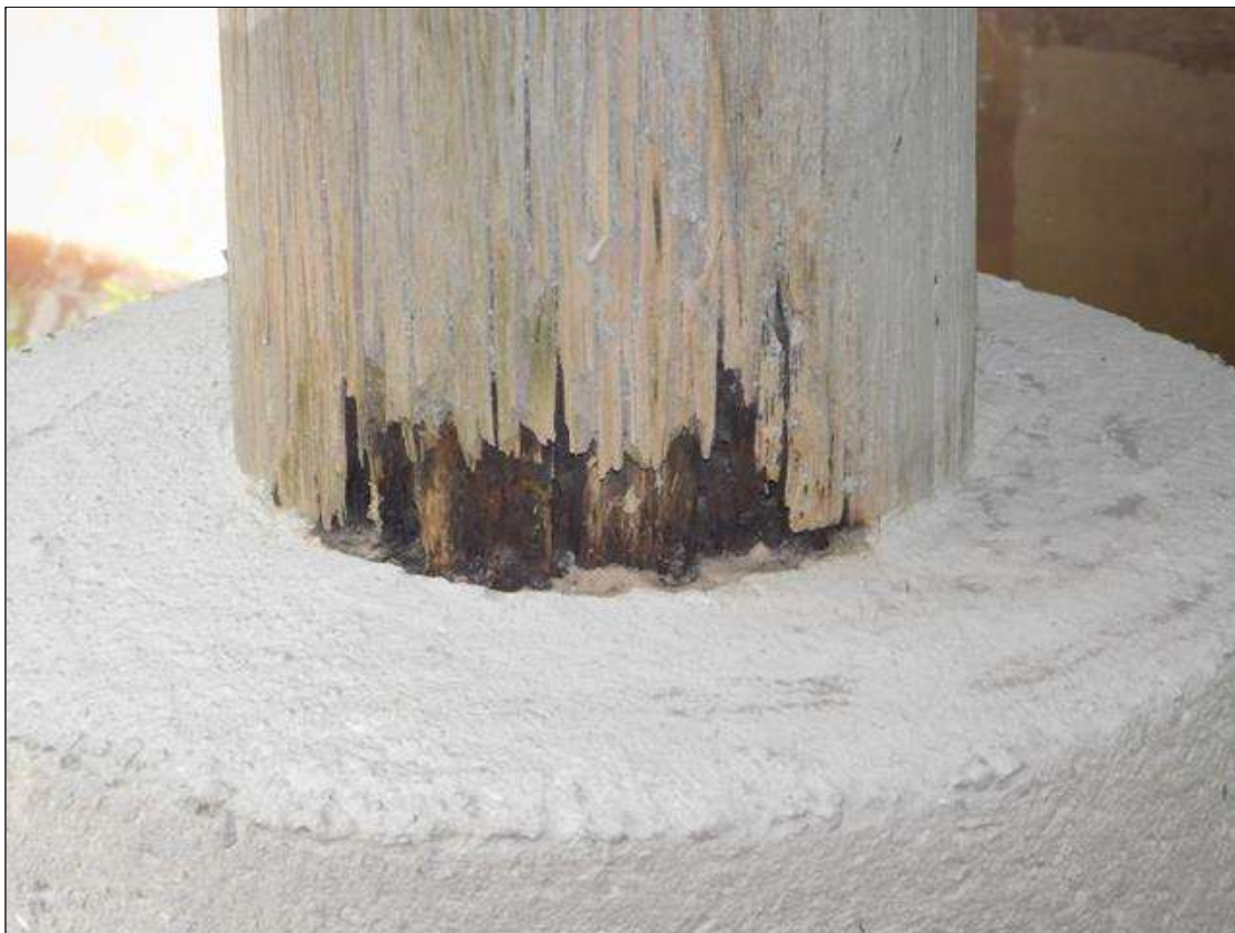
Bent 1 Pile 4: Northwest quadrant at top of collar, decay [7in x 4in x 3/4in]
