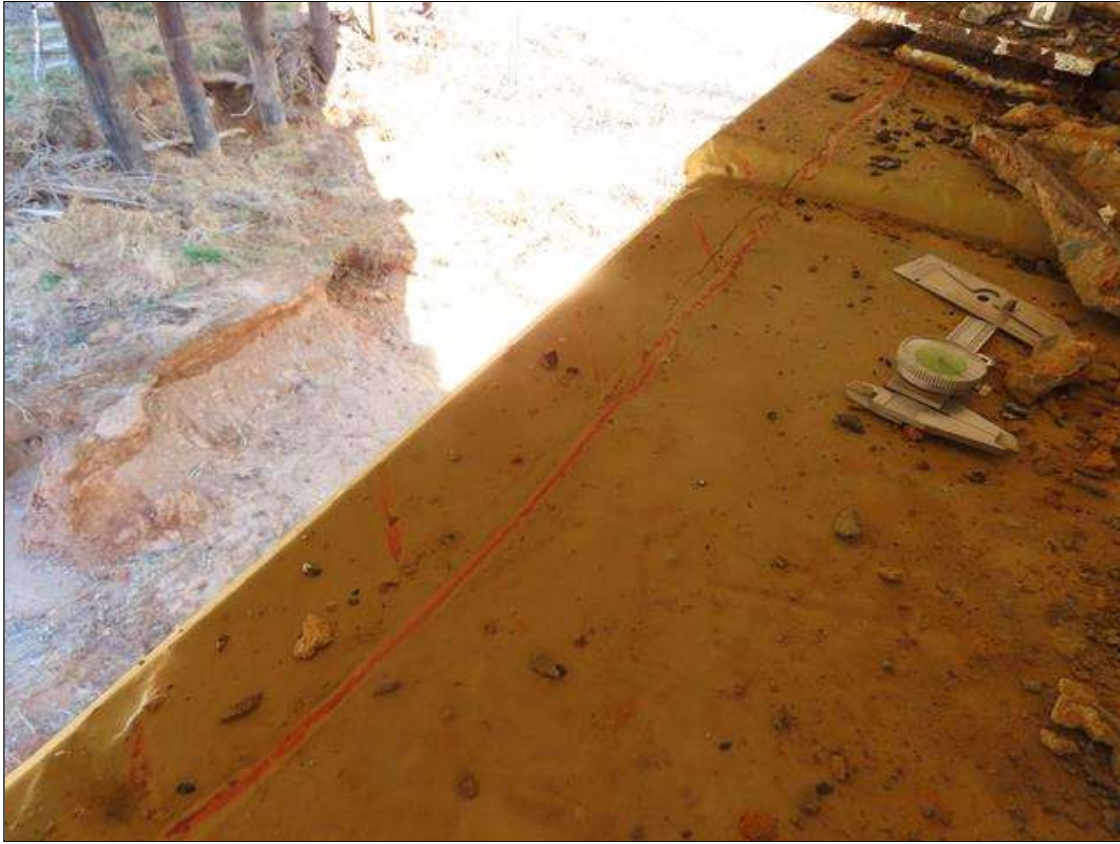
BENT 3 CAP - DELAM (4FT L. X 6IN W.) TO FAR SIDE TOP EDGE IN BAY 1 EXTENDING UP TO FAR EDGE OF SPAN 4 BEAM 2 NEAR END BEARING. (PAR)
