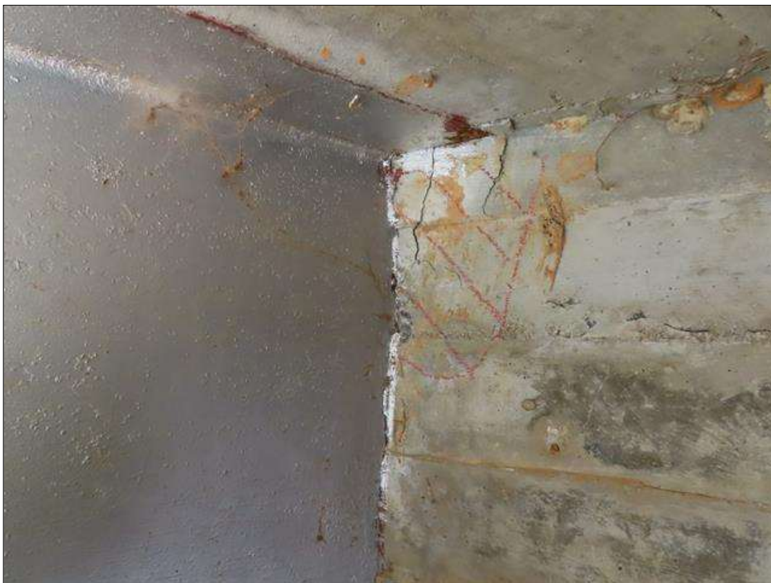
END BENT 1 ABUTMENT - DELAM (8IN L. X 5IN W.) TO BACKWALL AT LEFT SIDE OF BEAM 4. (SIMILAR AT LEFT SIDE OF BEAM 2)
