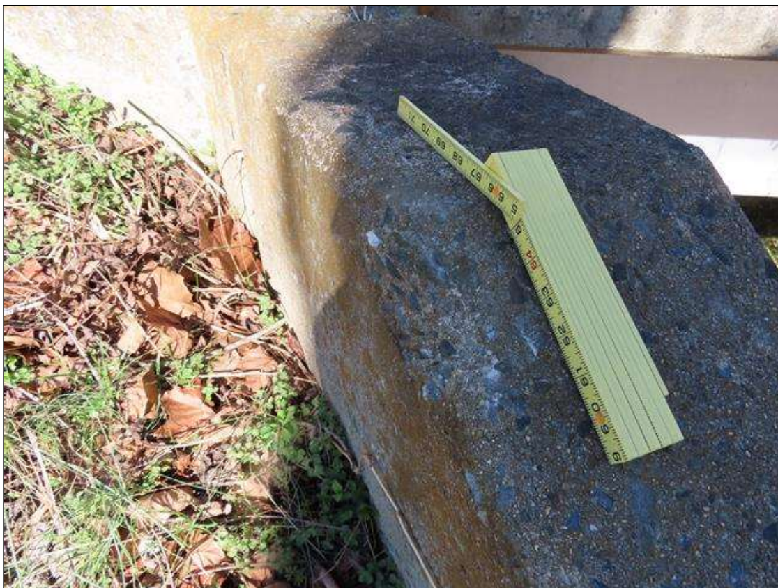
NEAR RIGHT (SW) WINGWALL - SPALL (5IN L. X 4IN W. X 1/2IN D.) TO NEAR SIDE AT TOP
