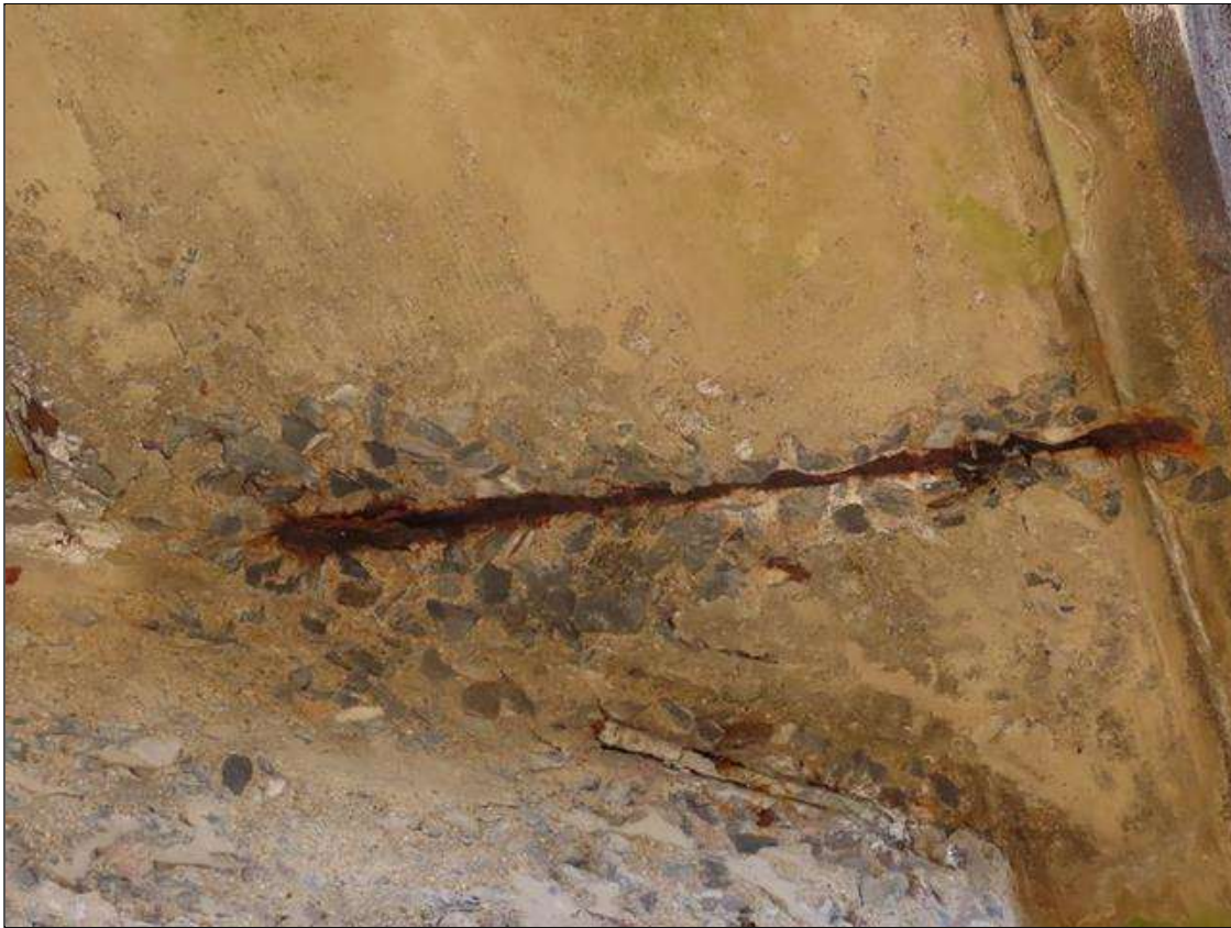
SPAN 1 DECK - SPALLING (18IN L. X 6IN W. X 1IN D.) WITH EXPOSED & CORRODED (1/16IN SL) REBAR TO BOTTOM OF RIGHT SIDE OVERHANG AT FAR END. (PAR)
