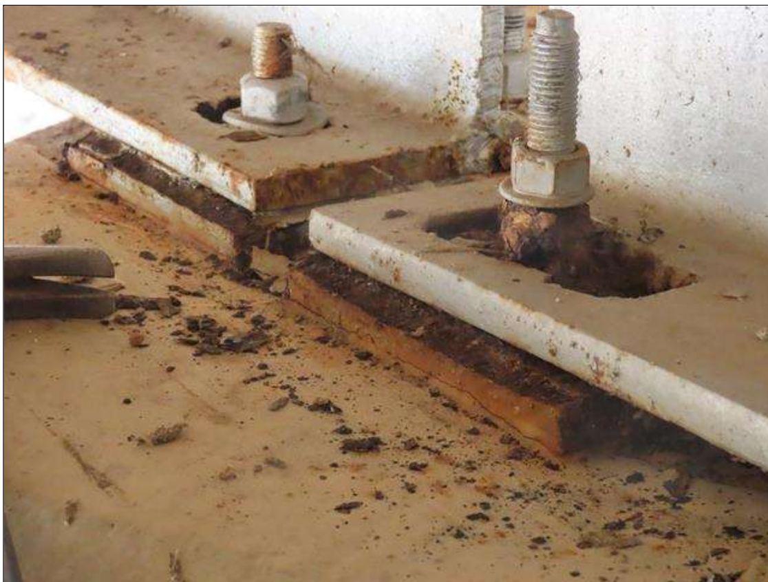
TYPICAL BEARINGS AT BENT 3, BEAMLINE 3 - MINOR TO MODERATE SCALE & CORROSION
