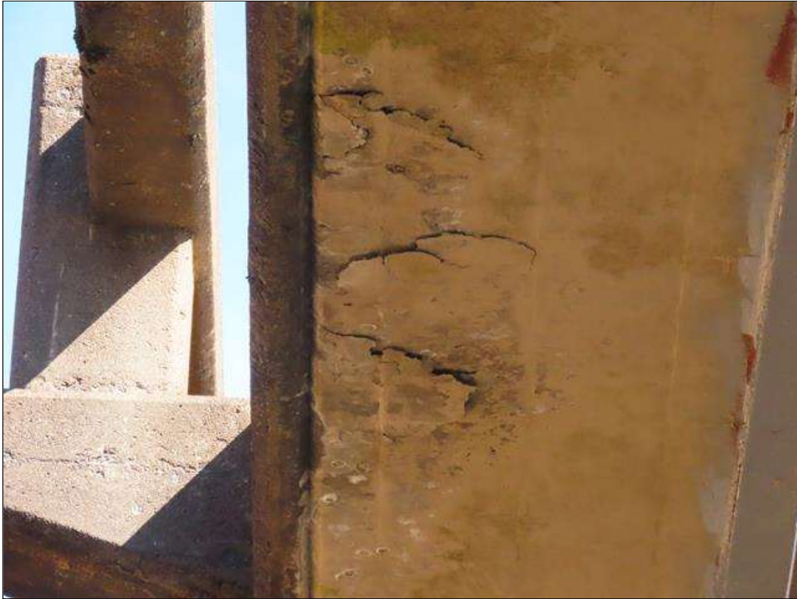
SPAN 3 DECK - DELAM (3SF) TO BOTTOM OF LEFT OVERHANG AT MID-SPAN
