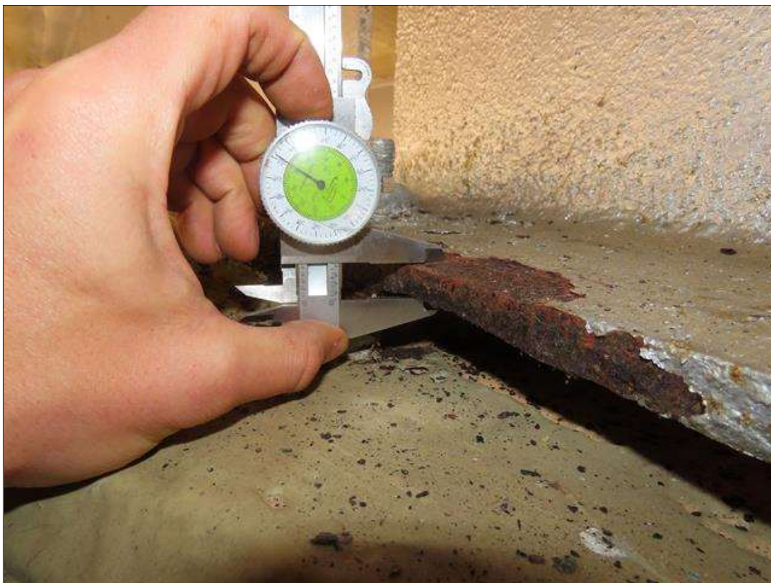
SPAN 2 BEAM 3 - BOTTOM FLANGE SECTION LOSS (UP TO 20%, 1/8IN SL, 1/2IN REMAIN) FULL W. FOR 1FT L. AT FAR END
