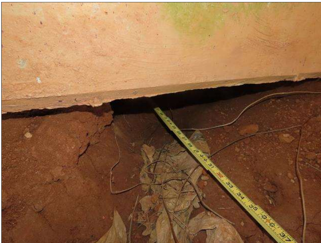
END BENT 2 CAP - EROSION UNDER CAP (UP TO 24IN D. X 3FT L.) BELOW BEAM 2. (PAR)
