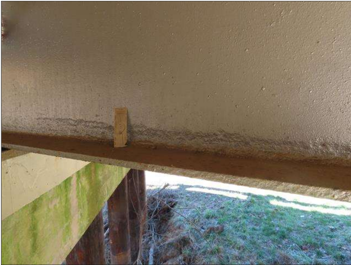
SPAN 5 BEAM 3 - ARRESTED WEB SECTION LOSS (UP TO 1/8IN SL, 3/8IN REMAIN) 2IN H. FOR 4FT L. TO BOTTOM AT NEAR END
