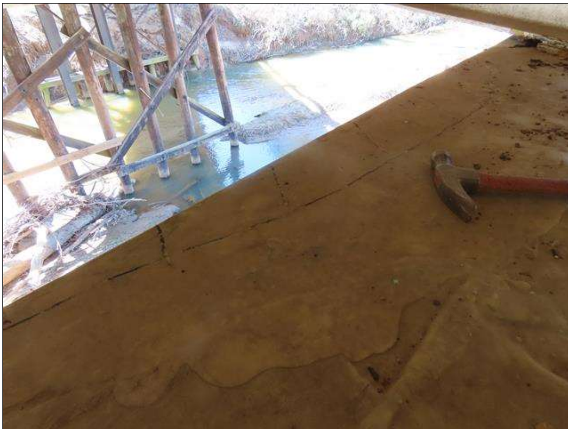
BENT 4 CAP - DELAM (3FT L. X 8IN W.) TO NEAR SIDE AT TOP EDGE IN BAY 1. (NOT UNDER BEARINGS)
