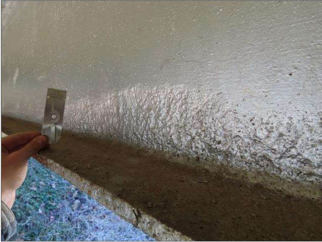
SPAN 1 BEAM 1 - ARRESTED WEB SECTION LOSS (UP TO 3/16IN SL, 5/16IN REMAIN) 4IN H. FOR 5FT L. TO BOTTOM RIGHT SIDE AT FAR END. (PAR)
