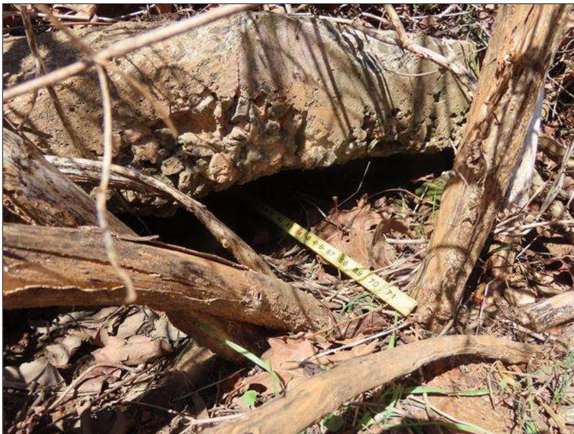
END BENT 2 SLOPE PROTECTION - EROSION UNDER CONCRETE SLOPE PROTECTION (6FT W. X 3FT L.) AT RIGHT SIDE. (PAR)
