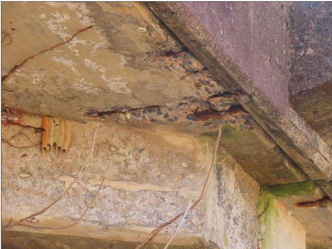
SPAN 3 DECK - SPALLING (2SF X 1IN D.) WITH EXPOSED & SCALING REBAR TO BOTTOM OF LEFT OVERHANG AT NEAR END
