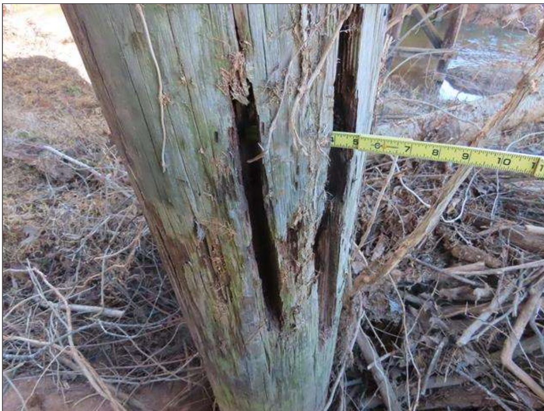
BENT 4 PILE 1 - DECAY/SECTION LOSS (UP TO 4IN D. X 12IN W. X 3FT L.) TO LEFT SIDE STARTING 2FT FROM GROUND. (PAR)
