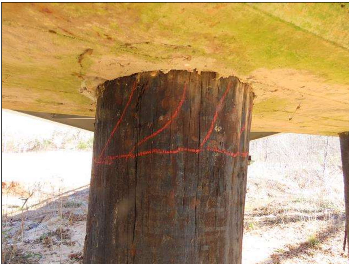
BENT 1 PILE 4 - HOLLOW WHEN SOUNDED (5IN H. X FULL PERIMETER) AT TOP. (PAR)
