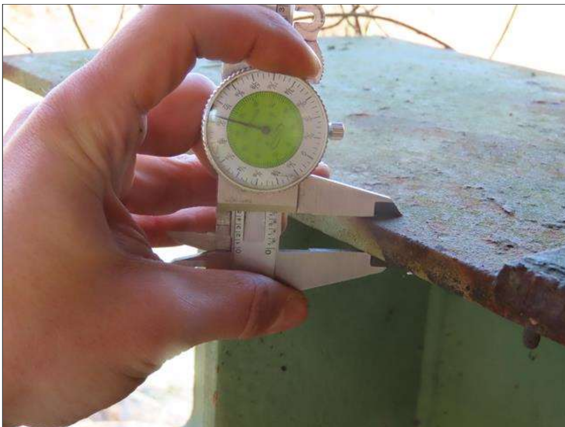
TYPICAL STEEL CAP FLANGE THICKNESS (7/16IN TH.) AT BENT 2, NEAR SIDE. (FAR SIDE STEEL CAP SIMILAR)
