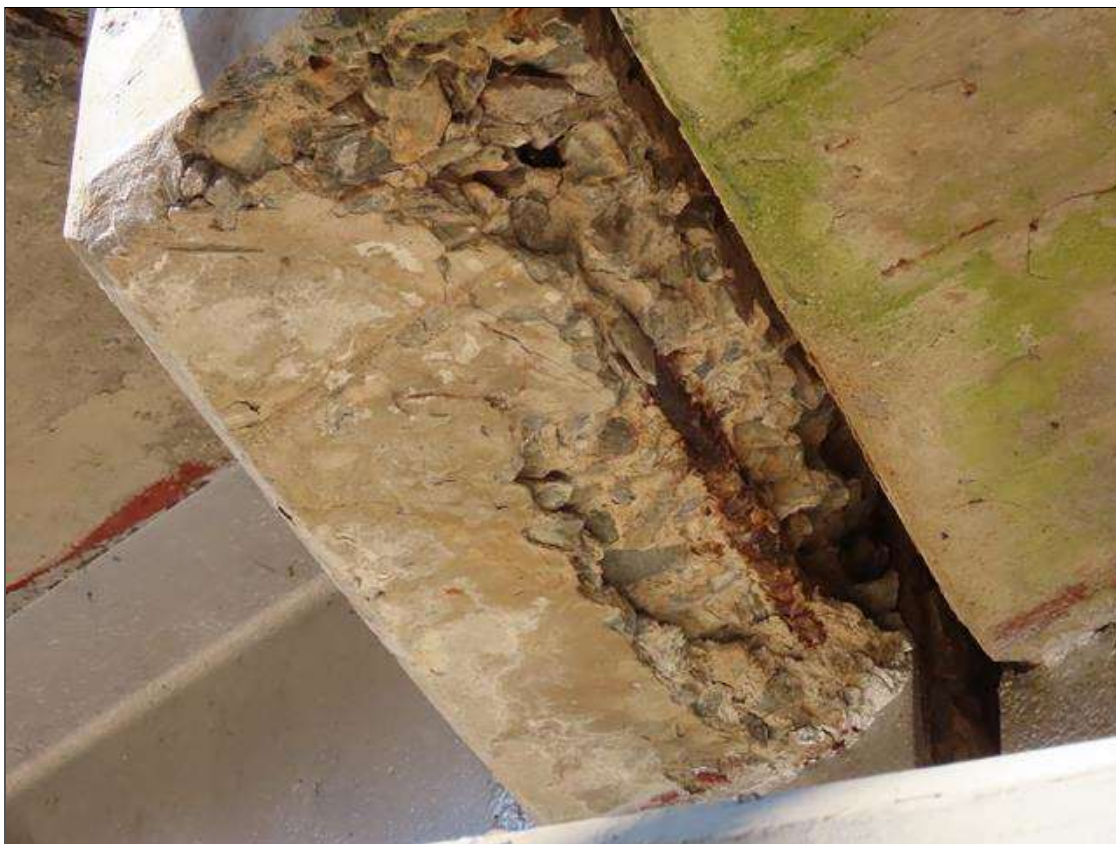
SPAN 1 BEAM 4, FAR END DIAPHRAGM - SPALL (2FT L. X 8IN W. X 2.5IN D.) WITH EXPOSED & CORRODED (1/16IN SL) REBAR AT RIGHT SIDE OF BEAM. (PAR)
