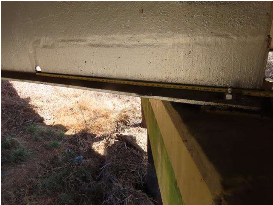
SPAN 5 BEAM 2 - BOTTOM FLANGE & WEB REPAIR (48IN L. X 6IN H.) AT NEAR END WITH 2IN DIAM. HOLE AT FAR END OF REPAIR
