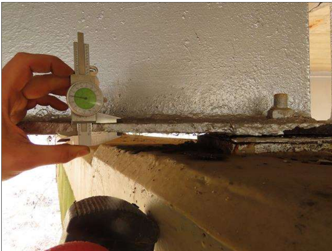
SPAN 5 BEAM 3 - BOTTOM FLANGE SECTION LOSS (UP TO 30%, 3/16IN SL, 7/16IN REMAIN) FULL W. FOR 6IN L. AT NEAR END. (PAR)
