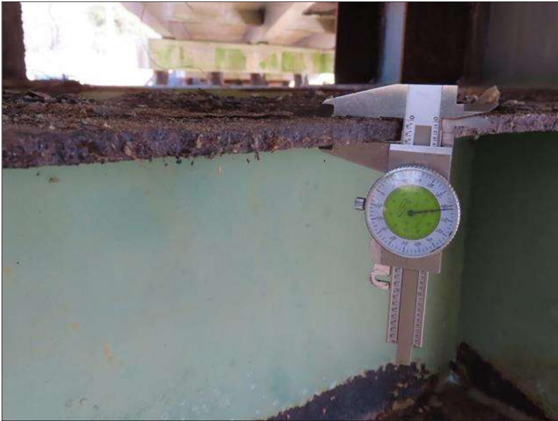
BENT 2 STEEL CAP, NEAR SIDE - TOP FLANGE SECTION LOSS (UP TO 1/16IN SL, 3/8IN REMAIN) FULL W. FOR 2.5FT L. BELOW BAY 1
