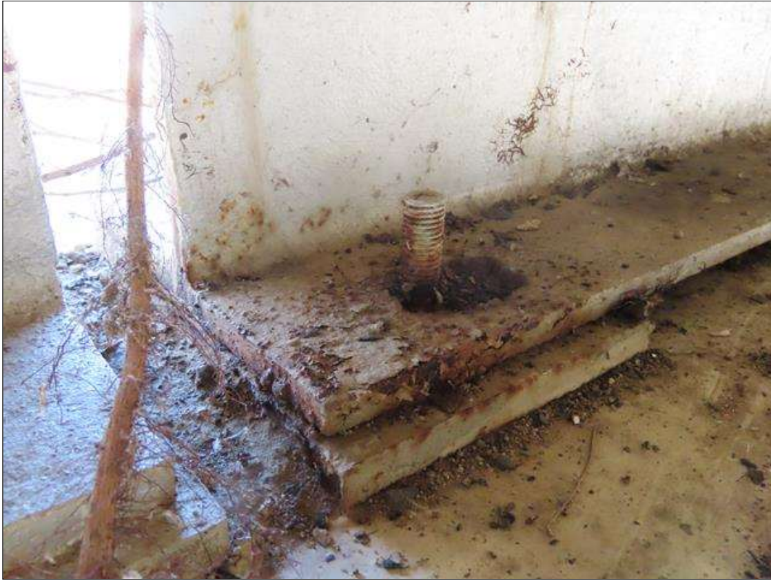
SPAN 3 BEAM 1, NEAR END BEARING - RIGHT ANCHOR NUT MISSING. (PAR)
