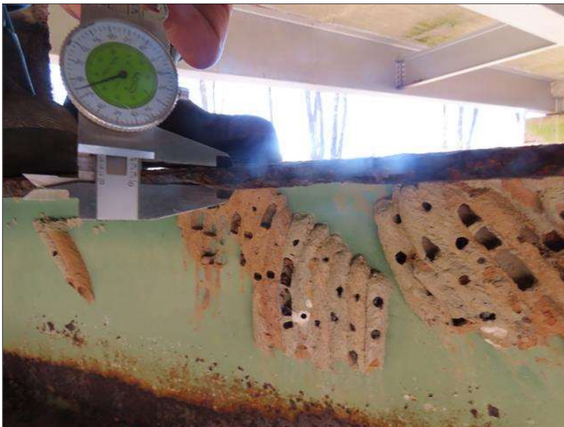
BENT 2 STEEL CAP AT NEAR SIDE - TAPERED TOP FLANGE SECTION LOSS (UP TO 1/8IN SL, 5/16IN REMAIN AT EDGE) FULL W. FOR 5FT L. BELOW BAY 2.
