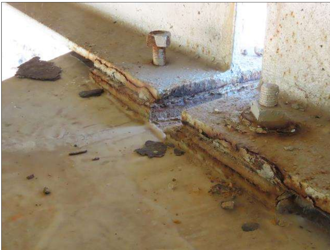
TYPICAL BEARINGS AT BENT 2, BEAMLIN 4 - MINOR TO MODERATE SCALE & CORROSION
