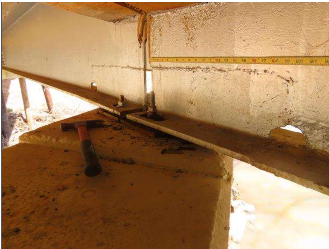
BEAMLINE 3 AT BENT 3 - BOTTOM FLANGE & WEB REPAIRS (20IN L. X 6IN H.) WITH 2IN DIAM. HOLE IN WEB AT END OF REPAIR.
