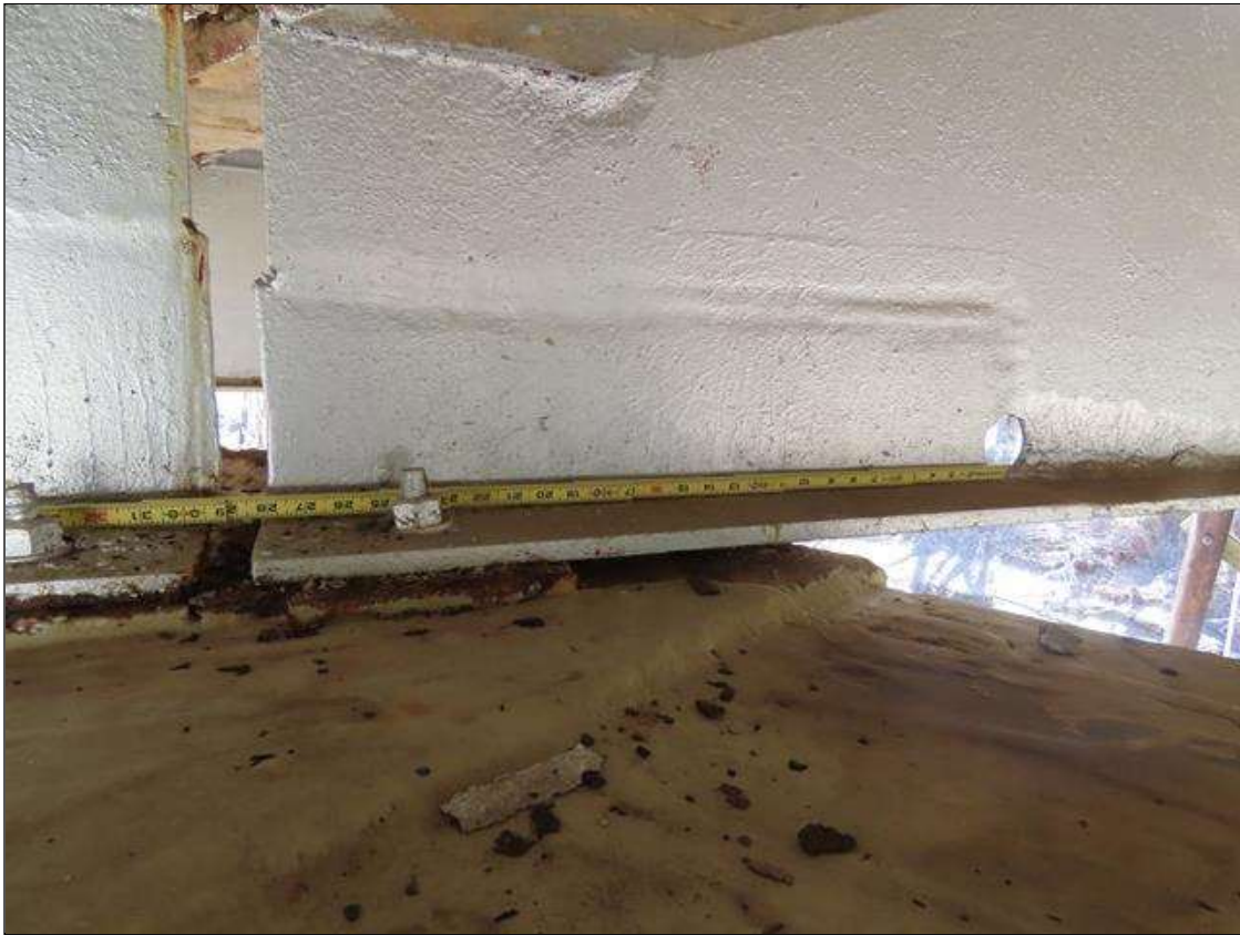
SPAN 4 BEAM 2 - BOTTOM FLANGE & WEB REPAIR (28IN L. X 6IN H.) AT FAR END WITH 2IN DIAM. HOLE IN WEB AT NEAR END OF REPAIR
