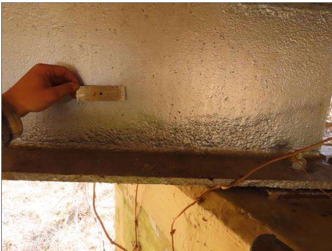
SPAN 5 BEAM 4 - ARRESTED WEB SECTION LOSS (UP TO 1/8IN SL, 3/8IN REMAIN) 3IN H. FOR 3FT L. TO BOTTOM AT NEAR END
