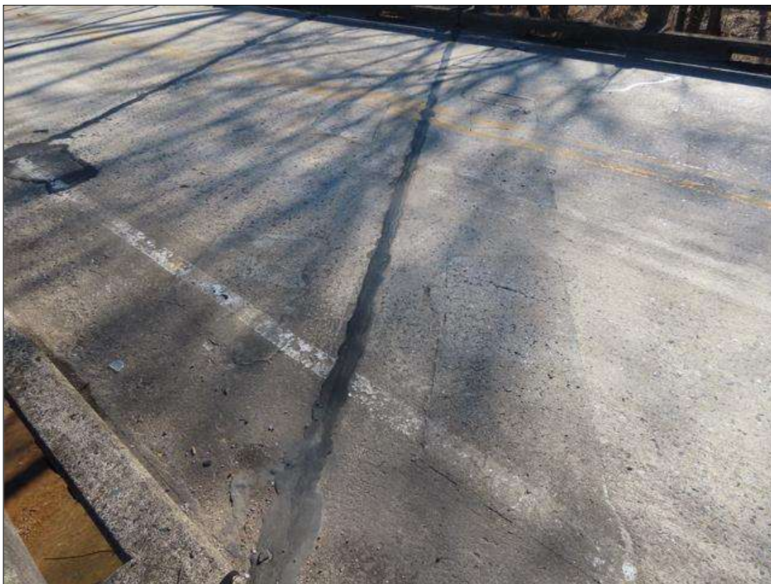
TYPICAL SOUND PATCHING (UP TO 5FT L. X 2FT W.) WITH HAIRLINE MAP CRACKING THROUGHOUT ENDS OF DECK ADJACENT TO JOINT OVER BENT 2
