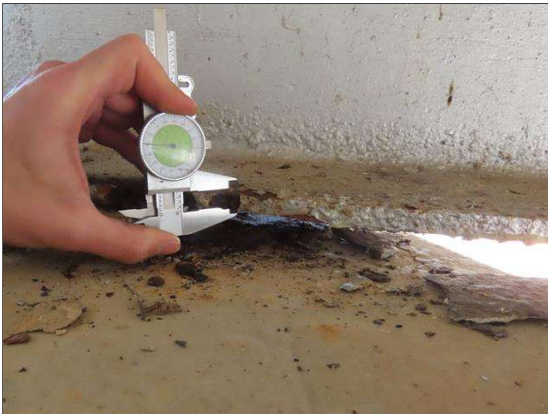
SPAN 4 BEAM 1 - BOTTOM FLANGE SECTION LOSS (UP TO 30%, 3/16IN SL, 7/16IN REMAIN) FULL W. FOR 6IN L. AT NEAR END. (PAR)
