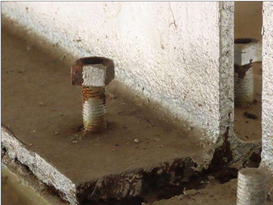
SPAN 3 BEAM 3, NEAR BEARING - BOTH ANCHOR NUTS NOT ENGAGED. (BEAM 2 & 4 AT NEAR END SIMILAR)
