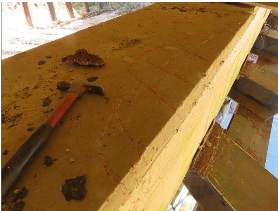
BENT 2 CAP - DELAM (3FT L. X 14IN W.) TO FAR SIDE TOP EDGE IN BAY 3. (NOT UNDER BEARING)
