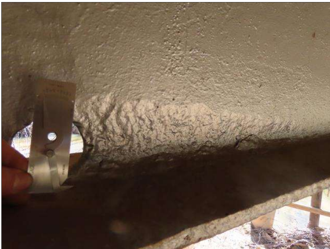
SPAN 4 BEAM 2 - ARRESTED WEB SECTION LOSS (UP TO 1/4IN SL, 1/4IN REMAIN) 2.5IN H. X 2FT L. STARTING 28IN FROM FAR END. (PAR)
