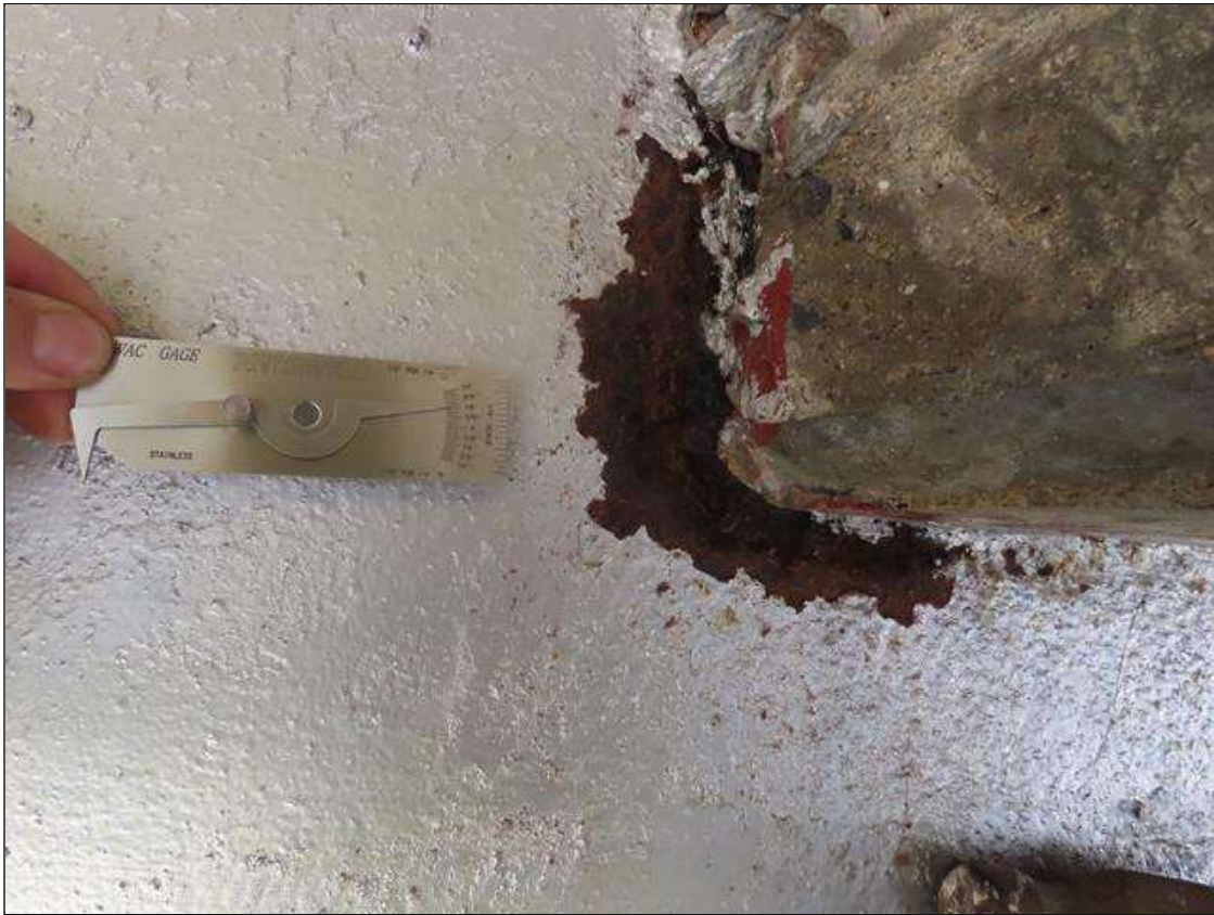
SPAN 1 BEAM 1 - WEB SECTION LOSS (UP TO 1/4IN SL, 1/4IN REMAIN) 1/8IN SL TO BOTH SIDES, 6IN L. X 1IN W. AT FAR END DIAPHRAGM. (PAR)
