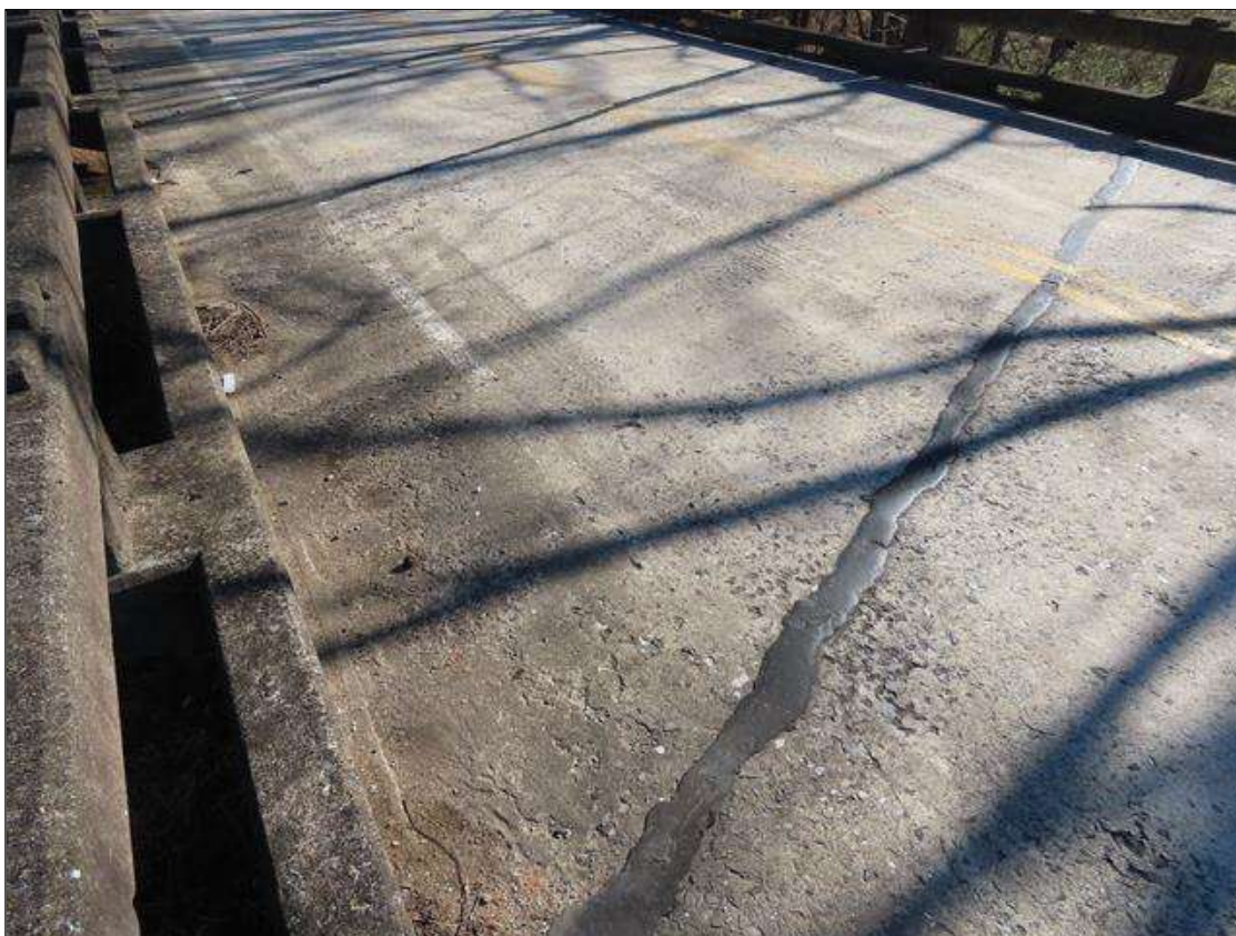
TYPICAL TRANSVERSE SEALED CRACKING (FULL W.) THROUGHOUT TOP OF DECK, SPAN 1 LOOKING AHEAD
