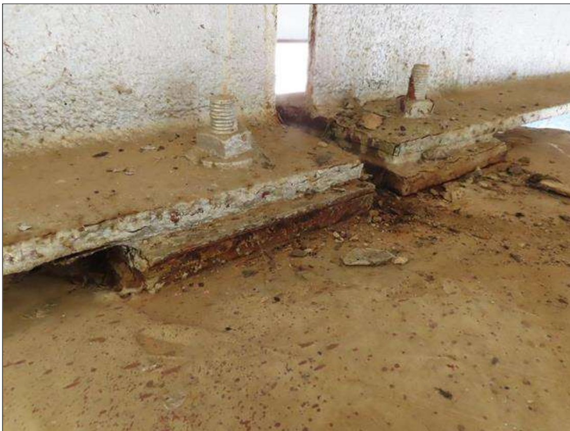
TYPICAL BEARINGS AT BENT 1, BEAMLIN 2 - MINOR SURFACE SCALE & CORROSION
