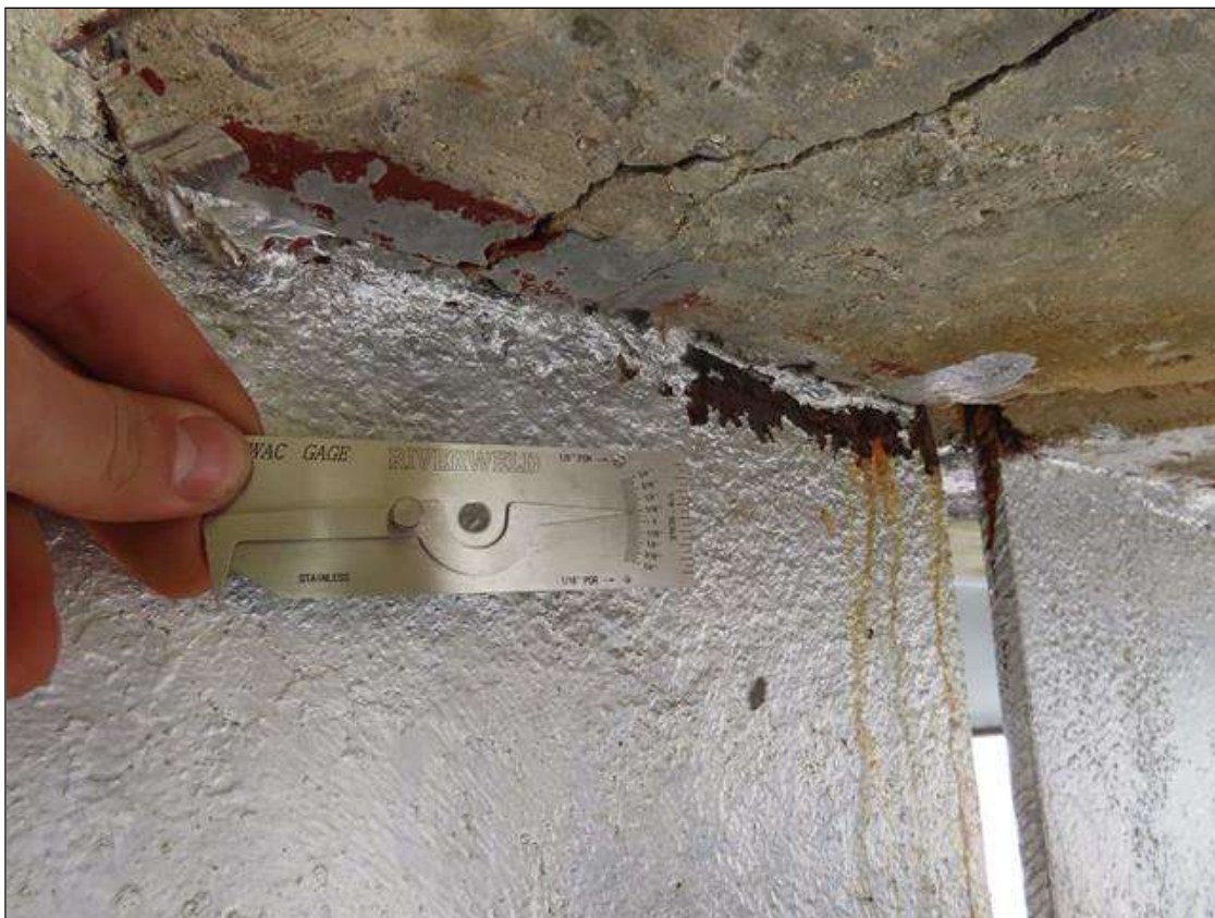
SPAN 1 BEAM 2 - WEB SECTION LOSS (UP TO 1/8IN SL, 3/8IN REMAIN) 1/16IN SL TO BOTH SIDES, 4IN L. X 1IN H. AT FAR END DIAPHRAGM. (PAR)
