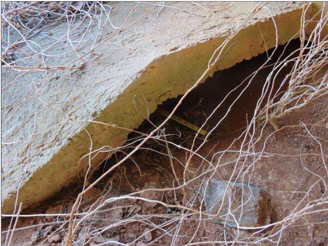
END BENT 2 SLOPE PROTECTION - EROSION UNDER CONCRETE SLOPE PROTECTION (6FT W. X 4FT L.) AT LEFT SIDE. (PAR PHOTO 2 OF 2)
