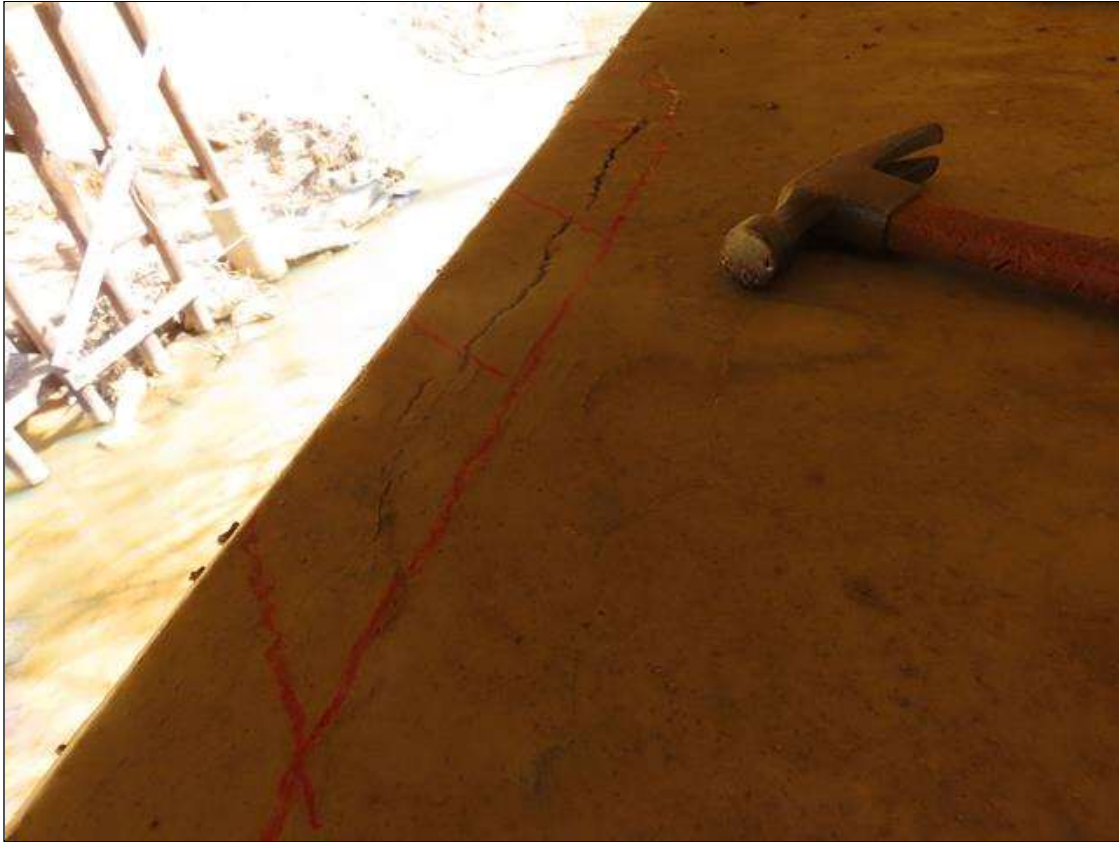
BENT 2 CAP - DELAM (4FT L. X 6IN W.) WITH 1/8IN OPEN CRACKING TO FAR SIDE AT TOP IN BAY 2. (NOT UNDER BEARING)
