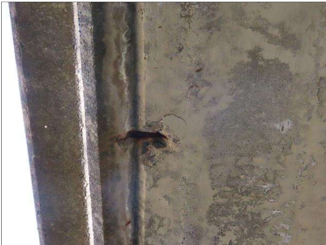
SPAN 1 DECK - SPALL (4IN DIAM. X 1/2IN D.) WITH EXPOSED REBAR TO BOTTOM OF LEFT OVERHANG AT MID-SPAN
