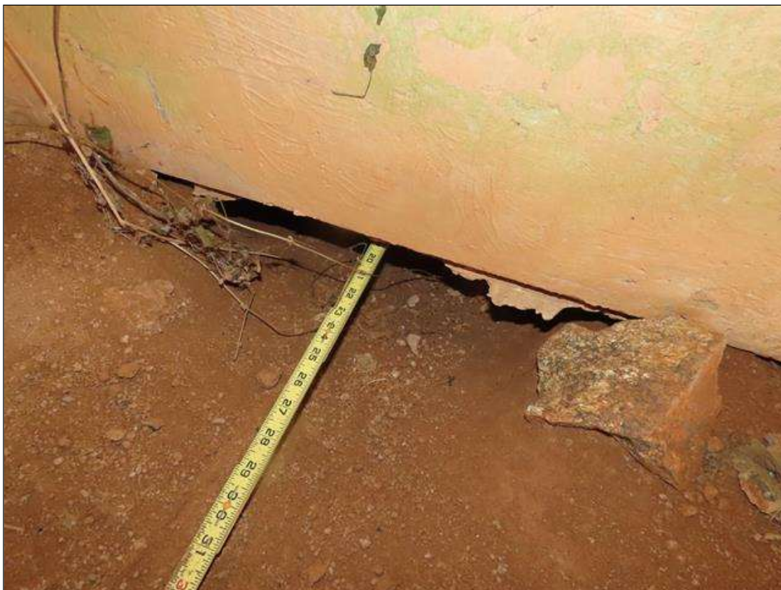
END BENT 2 CAP - EROSION UNDER CAP (UP TO 20IN D. X 2FT L.) BELOW BAY 1. (PAR)
