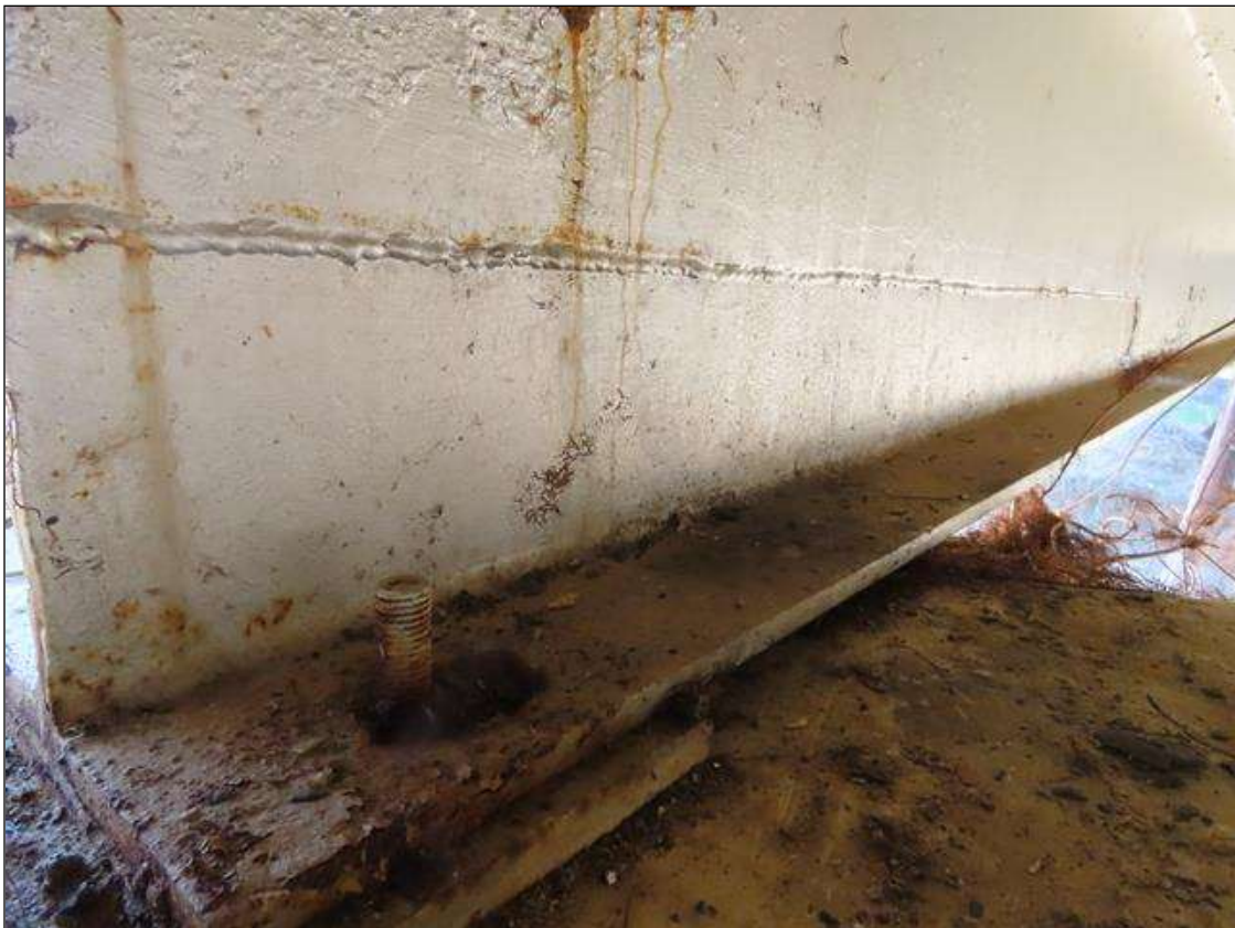
SPAN 3 BEAM 1 - BOTTOM FLANGE & WEB REPAIR (72IN L. X 6IN H.) AT NEAR END, WITH 2IN DIAM. HOLE AT FAR END OF REPAIR.
