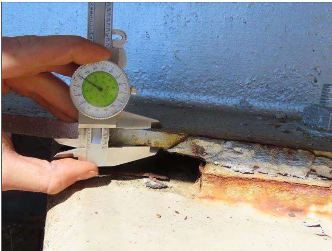
SPAN 2 BEAM 4 - BOTTOM FLANGE SECTION LOSS (UP TO 20%, 1/8IN SL, 1/2IN REMAIN) FULL W. FOR 6IN L. AT FAR END
