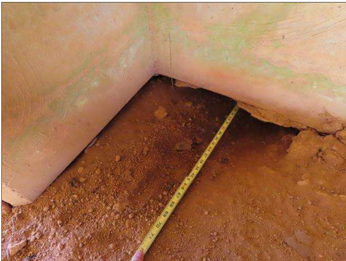
END BENT 1 CAP - EROSION UNDER CAP (2FT L. X 30IN D.) BELOW BAY 3. (PAR)
