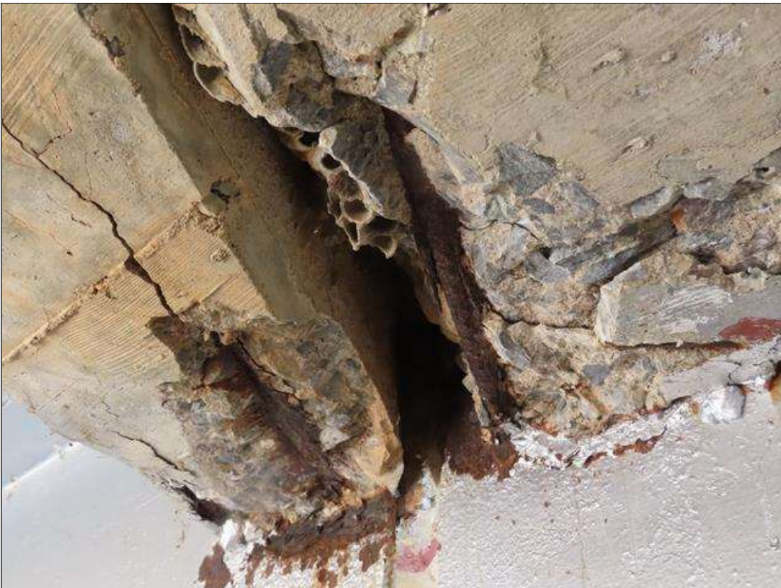
SPAN 3 & 4 DIAPHRAGMS AT BENT 3, BEAMLIN 2 - SPALLING (16IN L. X 6IN W. X 2IN D.) WITH EXPOSED & CORRODED (1/16IN SL) REBAR AT LEFT SIDE OF BEAMS (PAR)
