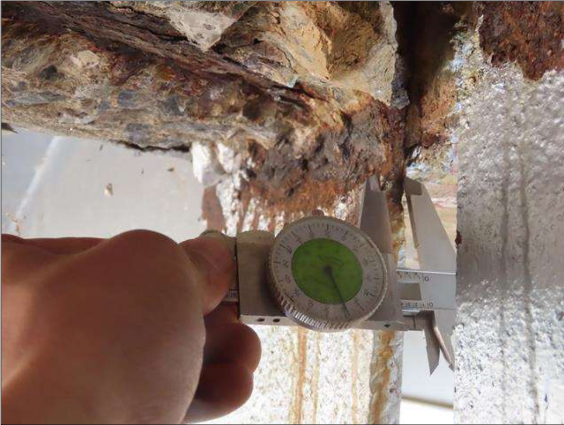
SPAN 4 BEAM 2 - WEB SECTION LOSS (UP TO 1/8IN SL, 3/8IN REMAIN) 6IN L. X 1IN H. AT NEAR END DIAPHRAGM. (PAR)
