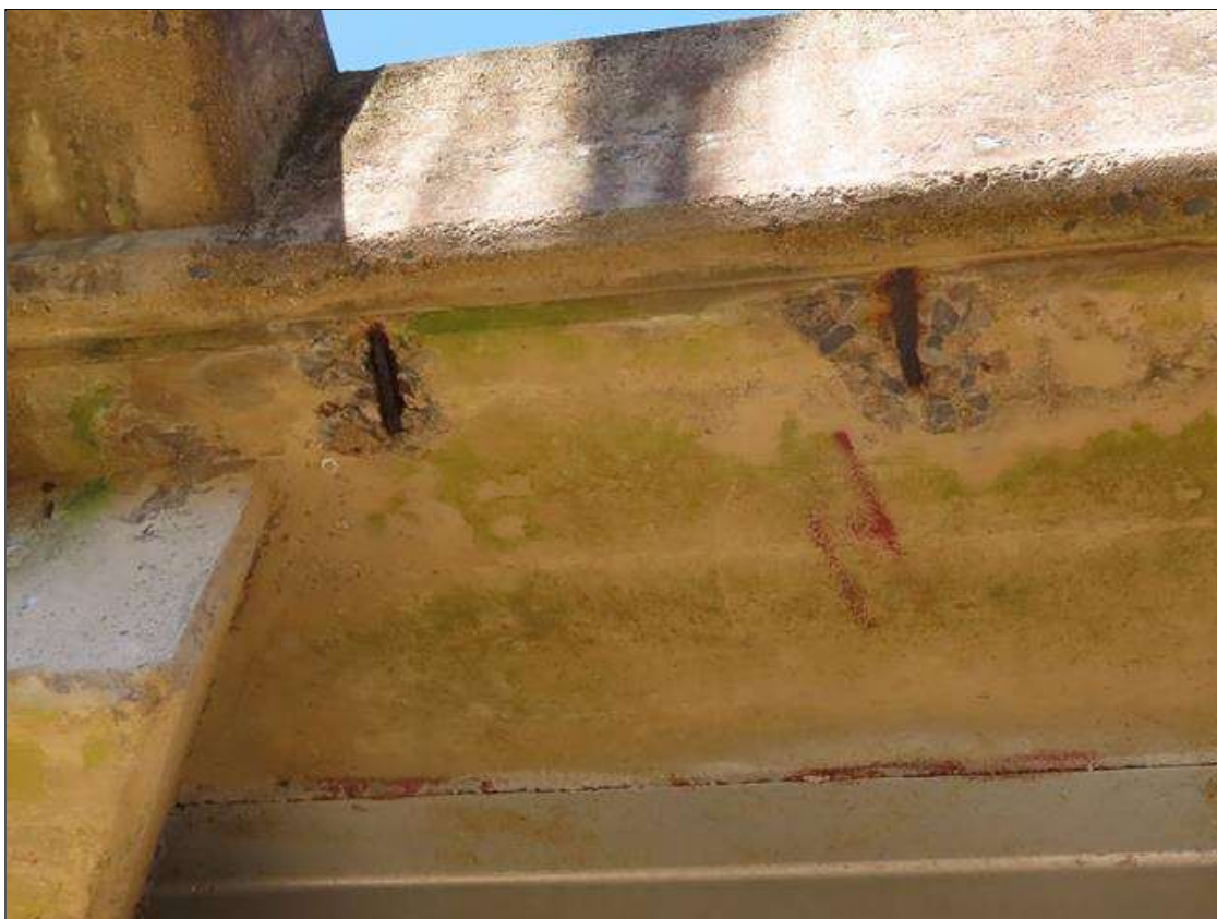
SPAN 2 DECK - X2 SPALLS (6IN DIAM. X 3/4IN D.) WITH EXPOSED & SCALING REBAR TO BOTTOM OF RIGHT SIDE OVERHANG AT NEAR END, (SIMILAR X2 AT FAR END).
