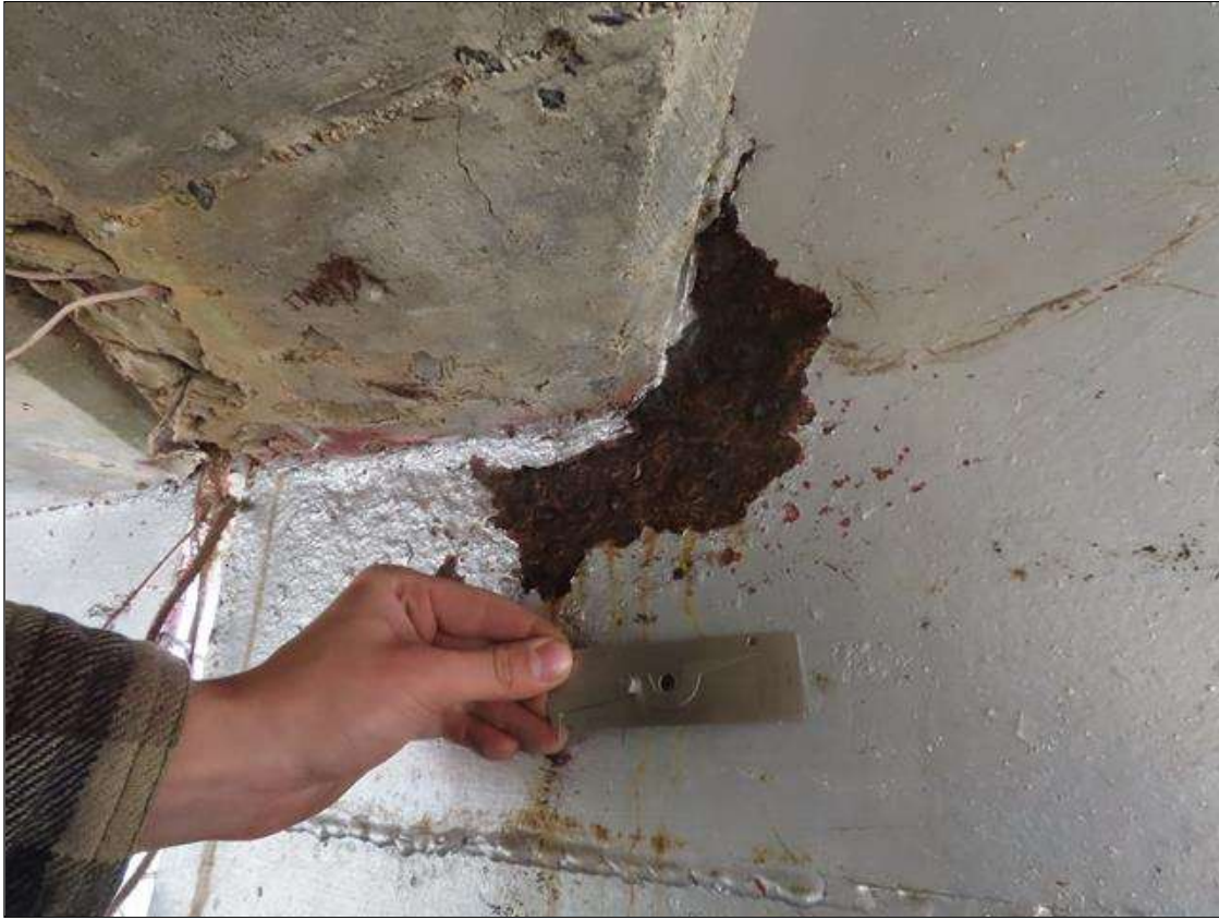
SPAN 3 BEAM 1 - WEB SECTION LOSS (UP TO 1/4IN SL, 1/4IN REMAIN) 3IN H. FOR 6IN H. AT NEAR END DIAPHRAGM. (PAR)
