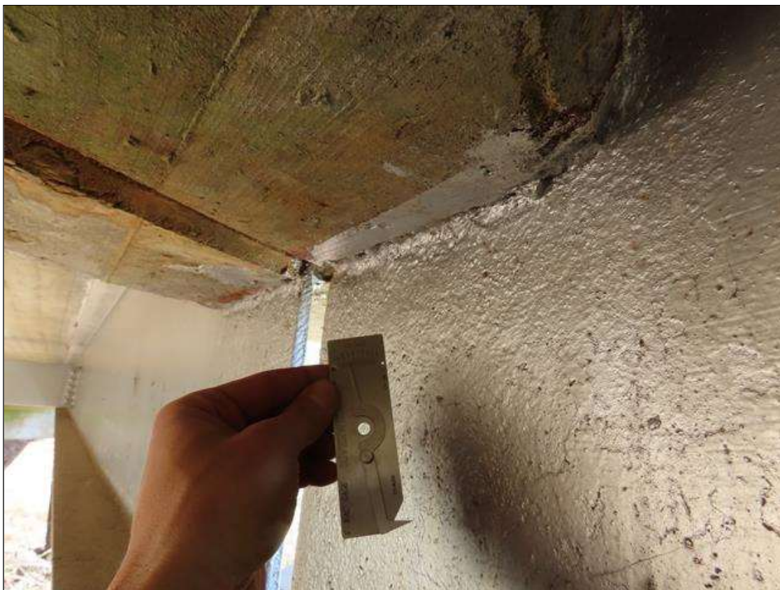
BEAMLINE 4 AT BENT 3 - ARRESTED WEB SECTION LOSS (UP TO 1/8IN SL, 3/8IN REMAIN) 6IN L. X 1IN H.) AT DIAPHRAGMS. (BEAMLINE 1 AT BENT 4 SIMILAR)
