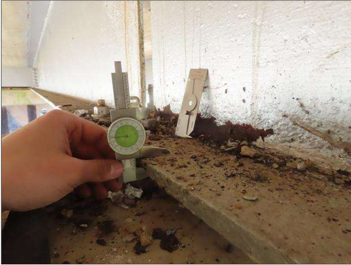
SPAN 3 BEAM 2 - BOTTOM FLANGE SECTION LOSS (UP TO 30%, 3/16IN SL, 7/16IN REMAIN) FULL W. FOR 6IN L. AT FAR END, AND WEB SECTION LOSS (UP TO 1/8IN SL, 3/8IN REMAIN) 12IN L. X 1IN H. TO BOTTOM AT FAR END, SIMILAR WEB SECTION LOSS AT TOP. (PAR)
