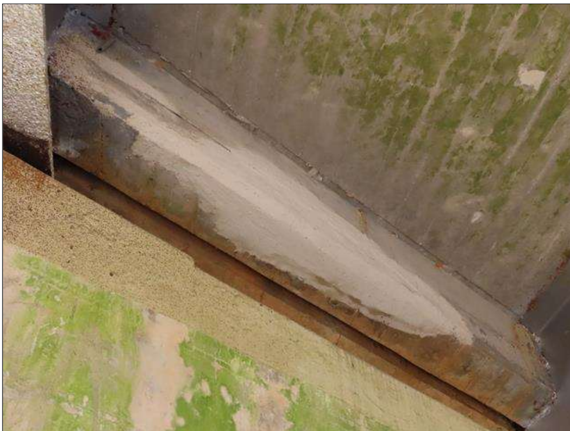
SPAN 2 BEAM 2, NEAR END DIAPHRAGM - SOUND PATCH (4FT L. X 10IN W.) AT RIGHT SIDE OF BEAM
