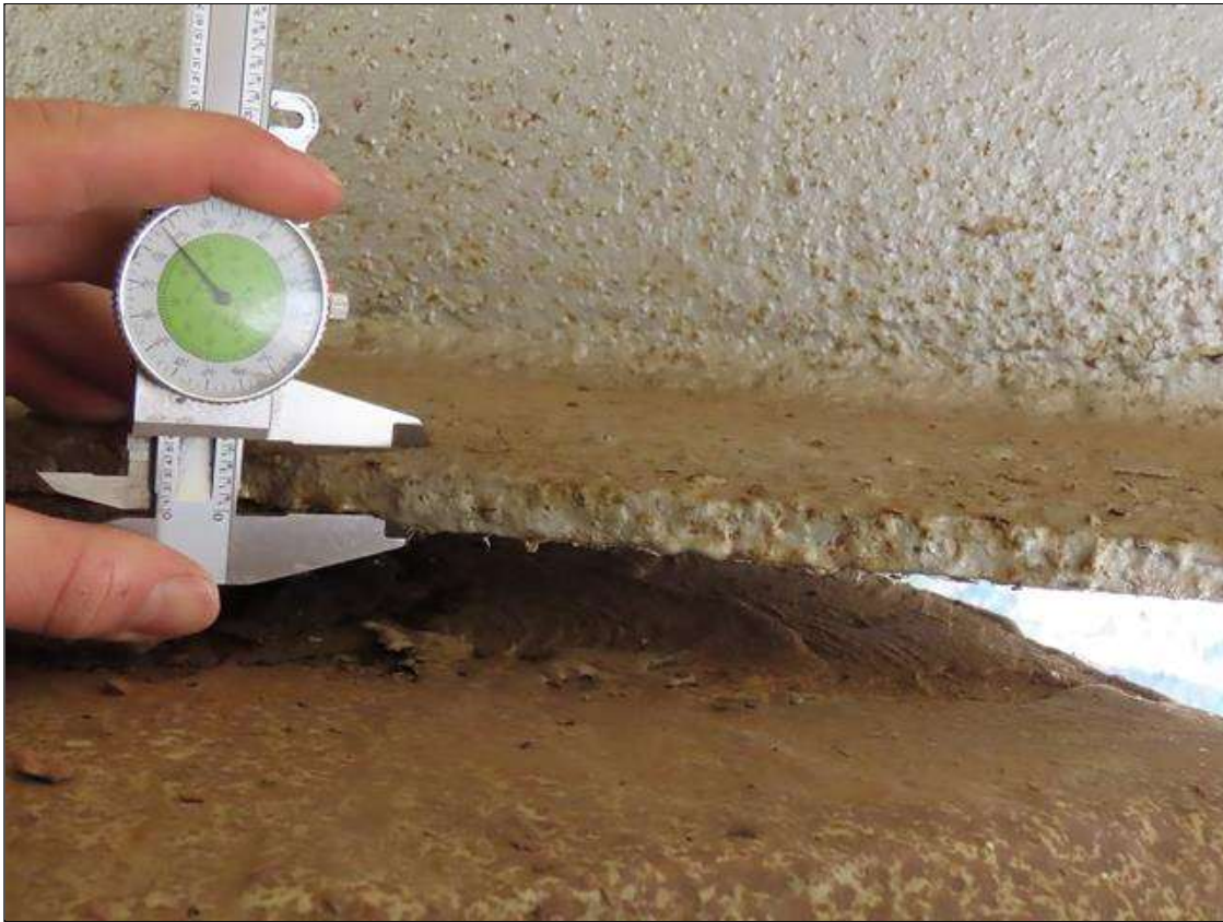
SPAN 2 BEAM 3 - ARRESTED BOTTOM FLANGE SECTION LOSS (UP TO 10%, 1/16IN SL, 9/1IN REMAIN) FULL W. FOR 16IN L. AT NEAR END
