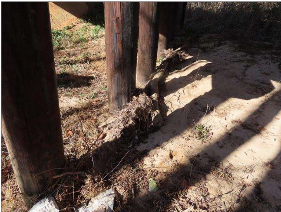
DRIFT (20FT L. X 2FT DIAM.) AT FAR SIDE OF BENT 1 AT GROUND
