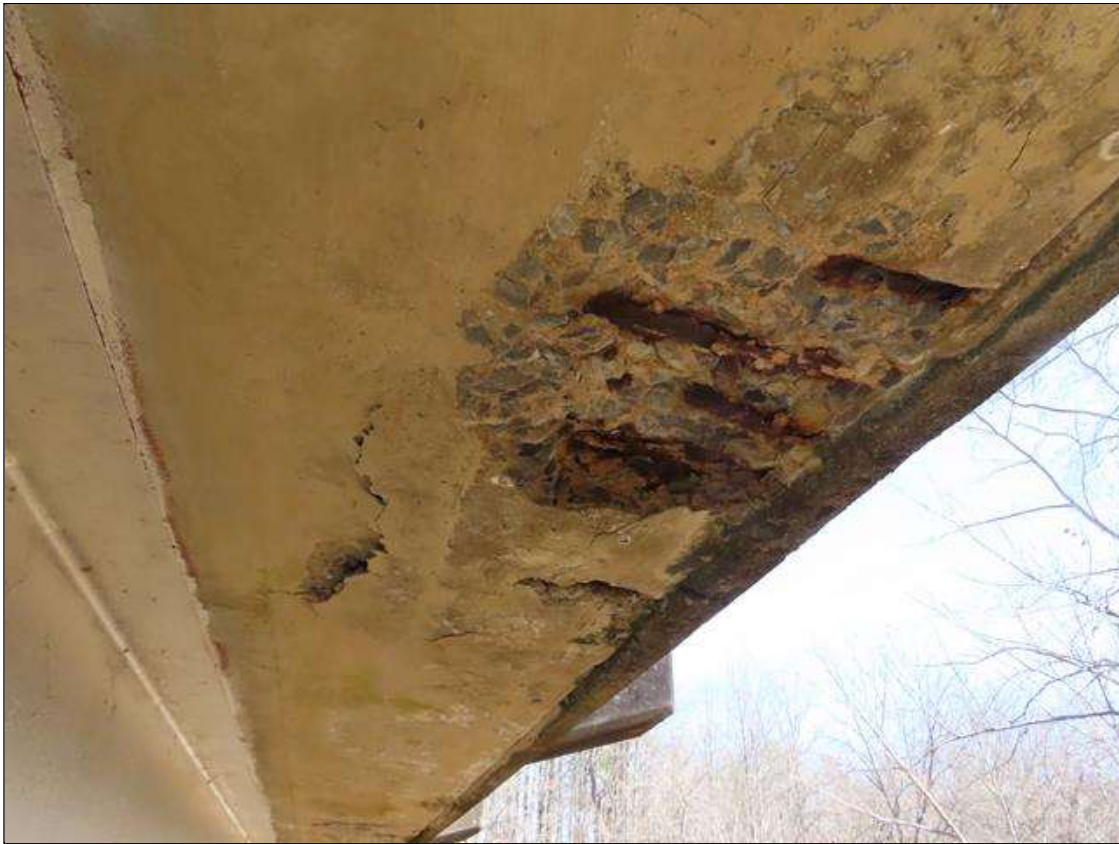
SPAN 3 DECK - SPALLING/DELAM (4.5FT L. X 14IN W. X 2IN D.) WITH EXPOSED & CORRODED (1/16IN SL) REBAR TO BOTTOM OF RIGHT OVERHANG, 2FT FROM NEAR END. (PAR)
