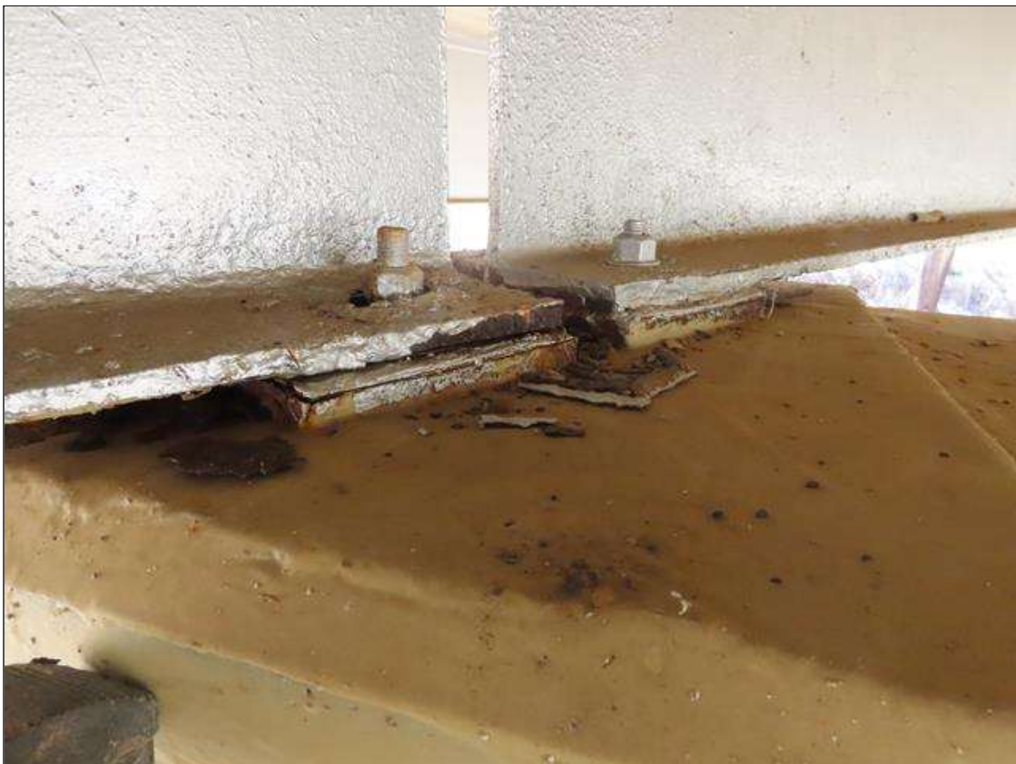
TYPICAL BEARINGS AT BENT 4, BEAMLIN 3 - MINOR TO MODERATE SCALE & CORROSION
