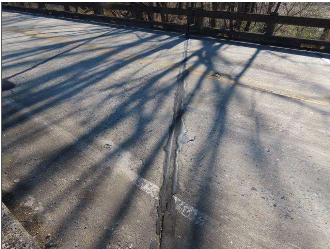
JOINT OVER BENT 1 - INTERMITTENT CRACKING (UP TO 1/4IN W.) THROUGHOUT SEAL
