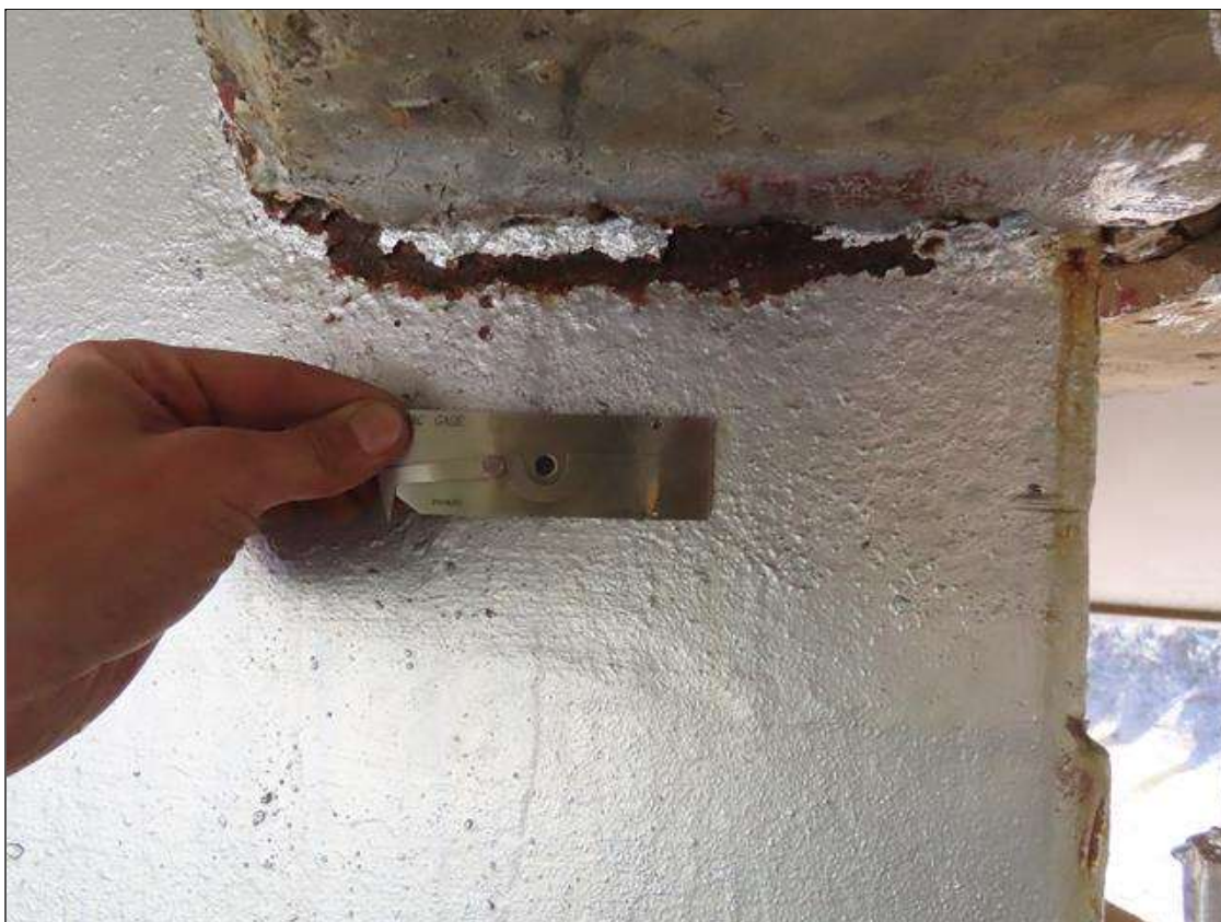
SPAN 5 BEAM 2 - WEB SECTION LOSS (UP TO 1/8IN SL, 3/8IN REMAIN) 6IN L. X 1IN H. AT NEAR END DIAPHRAGM. (PAR)
