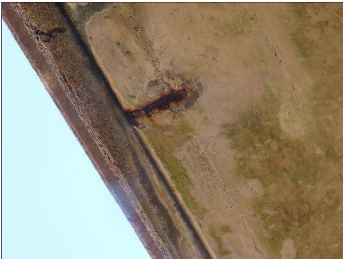
SPAN 2 DECK - SPALL (6IN DIAM. X 1/2IN D.) WITH EXPOSED REBAR TO BOTTOM OF LEFT OVERHANG 10FT FROM NEAR END
