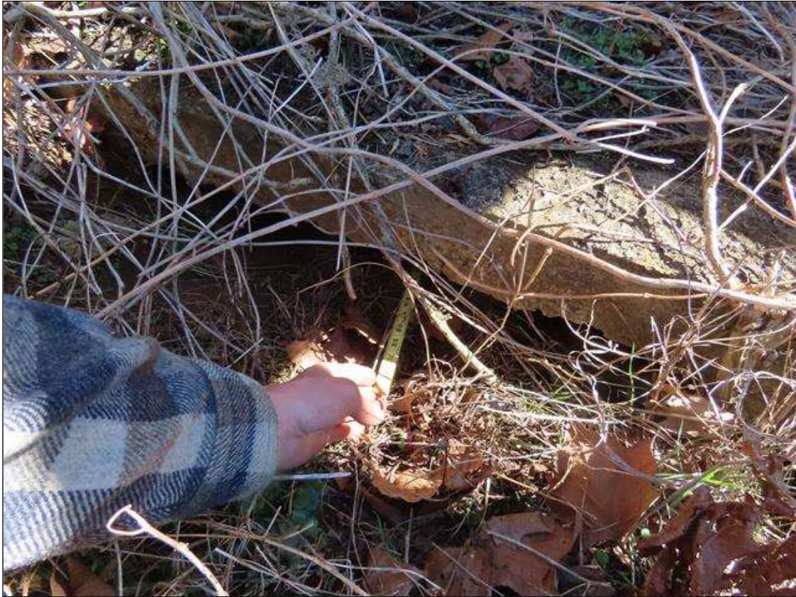
END BENT 2 SLOPE PROTECTION - EROSION UNDER CONCRETE SLOPE PROTECTION (6FT W. X 4FT L.) AT LEFT SIDE. (PAR PHOTO 1 OF 2)
