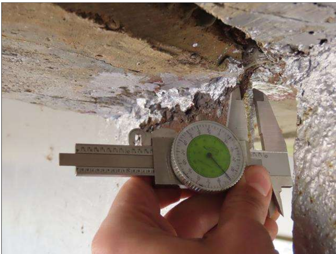
SPAN 3 BEAM 3 - WEB SECTION LOSS (UP TO 3/16IN SL, 5/16IN REMAIN) 6IN L. X 1IN H. AT NEAR END DIAPHRAGM. (PAR)
