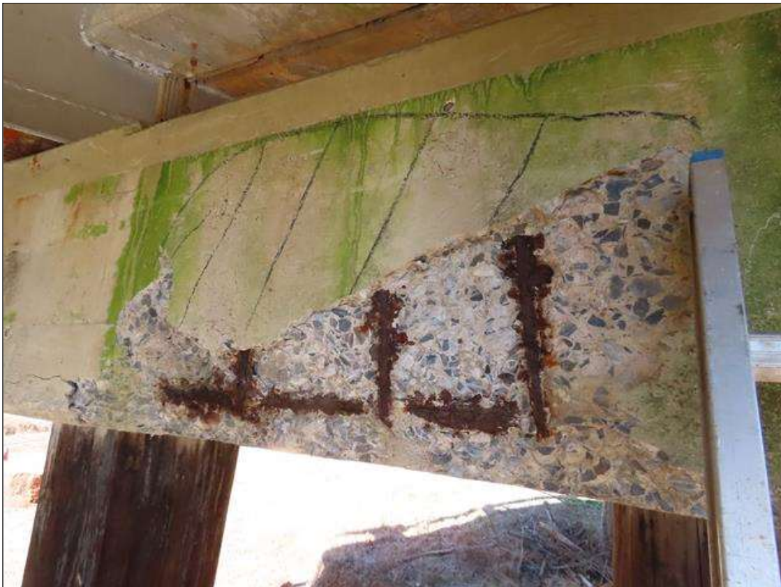
BENT 3 CAP - SPALLING/DELAM (40IN L. X 24IN . X 2IN D.) WITH EXPOSED & CORRODED (1/16IN SL) REBAR TO NEAR SIDE BELOW BAY 3. (PAR)
