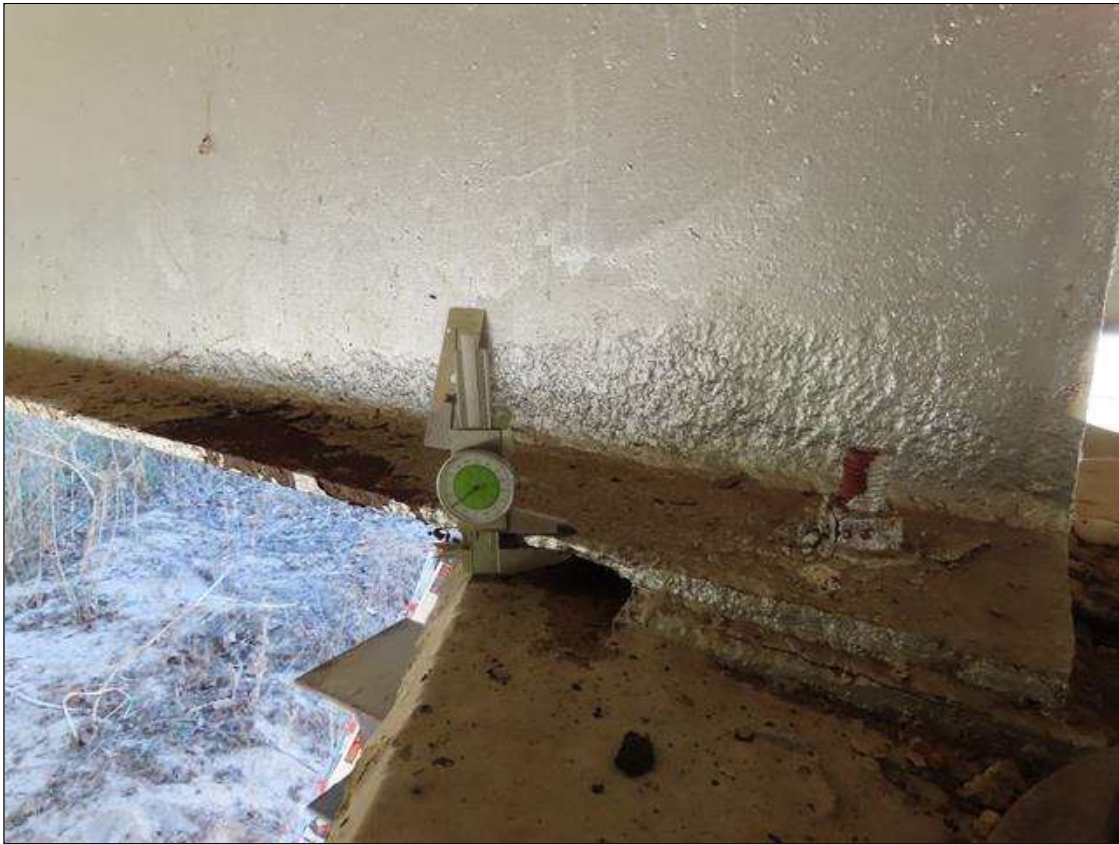
SPAN 2 BEAM 2 - TAPERED BOTTOM FLANGE SECTION LOSS (UP TO 15%, 5/16IN SL, 5/16IN REMAIN AT EDGE) 6IN W. FOR 1FT L. AND ARRESTED WEB SECTION LOSS (UP TO 3/16IN SL, 5/16IN REMAIN) 4IN H. X 2FT L. TO BOTTOM AT FAR END. (PAR)
