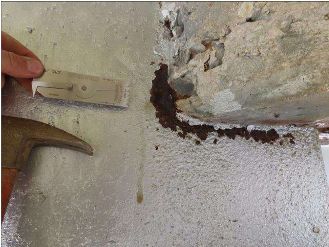
SPAN 1 BEAM 3 - WEB SECTION LOSS (UP TO 1/8IN SL, 3/8IN REMAIN) 6IN L. X 1IN W. AT FAR END DIAPHRAGM. (PAR)
