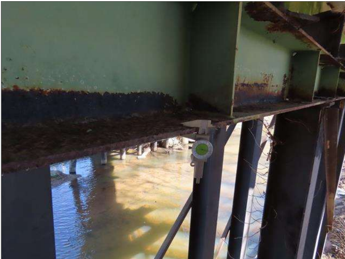
TYPICAL INTERMITTENT MODERATE TO HEAVY SCALE & CORROSION, NO MEASURABLE SECTION LOSS, THROUGHOUT STEEL CAP & BEAMS AT BENT 2, NEAR SIDE BELOW BEAM 2
