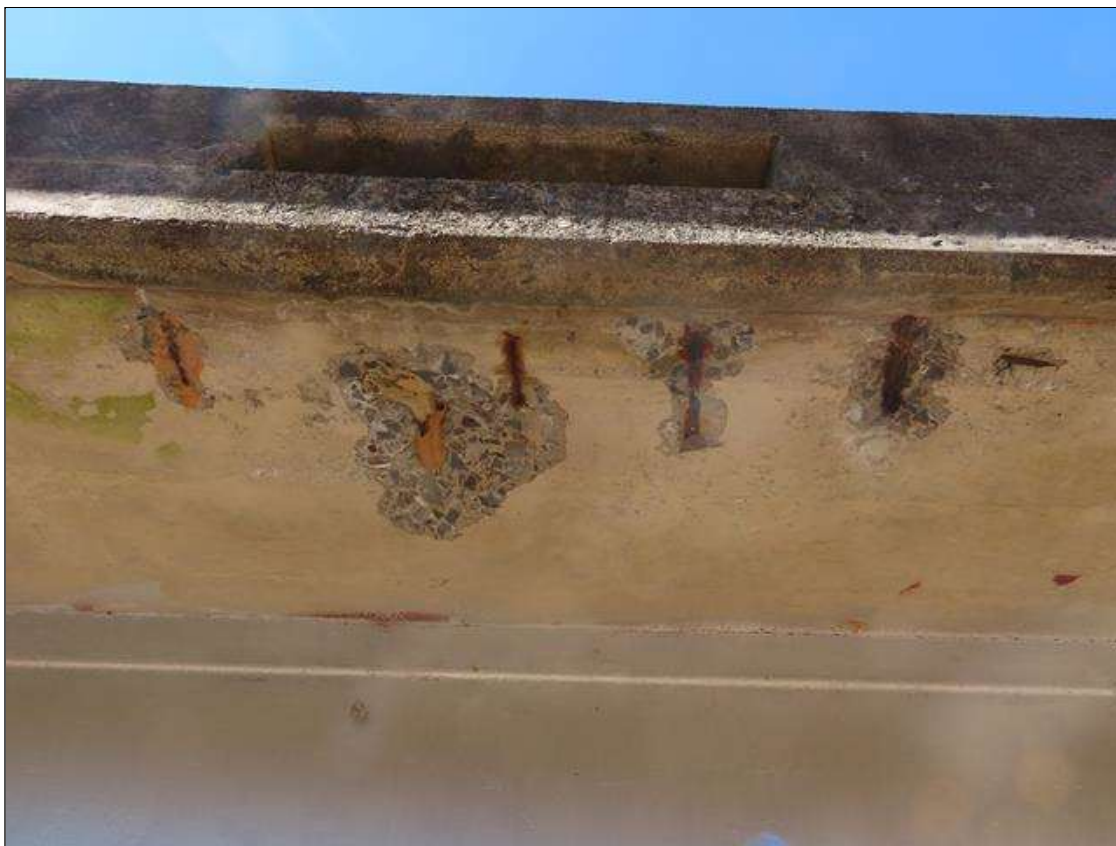
SPAN 5 DECK - SPALLING (UP TO 12IN DIAM. X 1IN D.) WITH EXPOSED & CORRODED (1/16IN SL) REBAR TO BOTTOM OF RIGHT SIDE OVERHANG 10FT FROM END BENT 2. (PAR)
