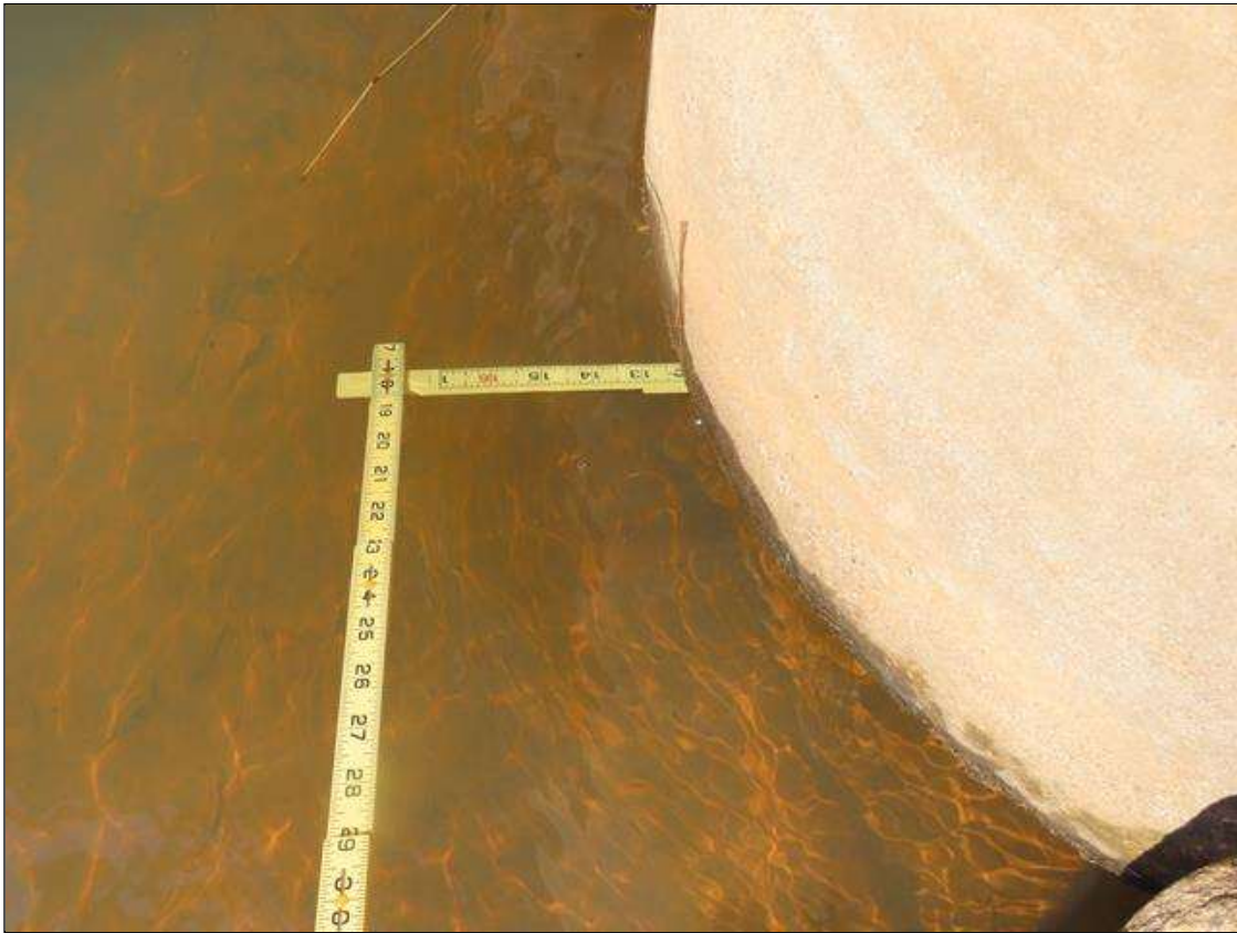
BENT 3 PILE 7 - SCOUR (UP TO 1.1FT D.) AT CONCRETE COLLAR WITH UNDERMINE TO COLLAR (UP TO 12IN D. X 1/2 PERIMETER) AT NEAR SIDE
