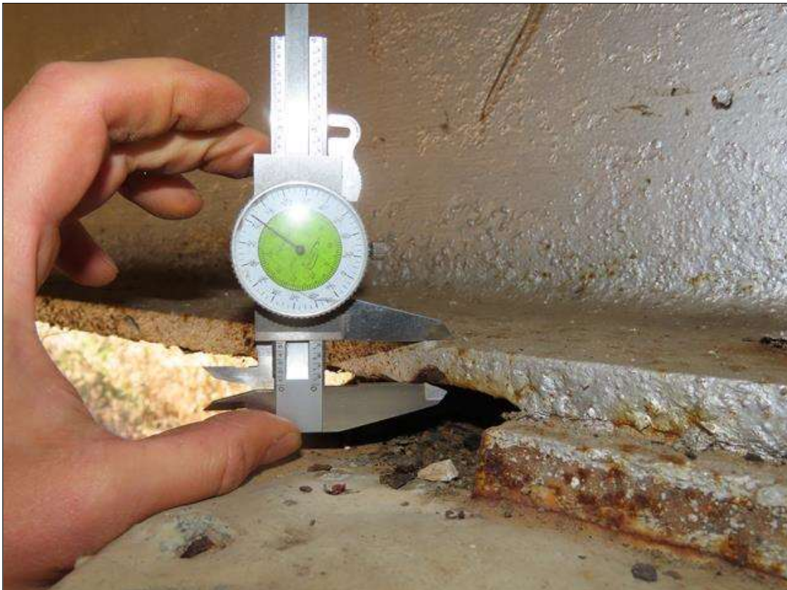
SPAN 2 BEAM 1 - BOTTOM FLANGE SECTION LOSS (UP TO 20%, 1/8IN SL, 1/2IN REMAIN) FULL W. FOR 1FT L. AT FAR END
