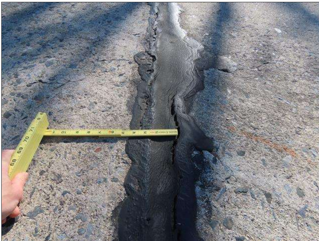
TYPICAL AREA OF CRACKING (UP TO 1/4IN W.) THROUGHOUT SEAL, JOINT OVER BENT 1 LEFT LANE
