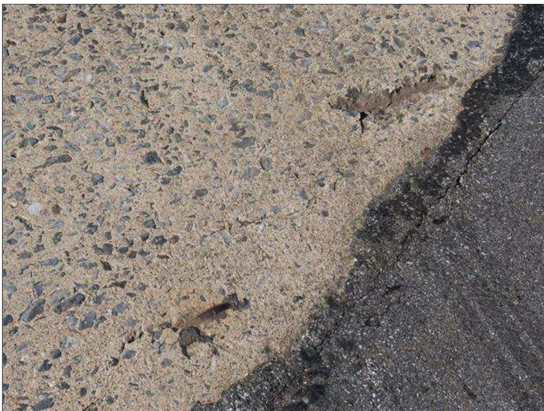
TYPICAL INTERMITTENT SPALLING/DELAM (UP TO 12IN L. X 5IN W. X 1/2IN D.) WITH EXPOSED REBAR TO TOP OF DECK THROUGHOUT FAR END, RIGHT LANE SHOWN. (PAR)
