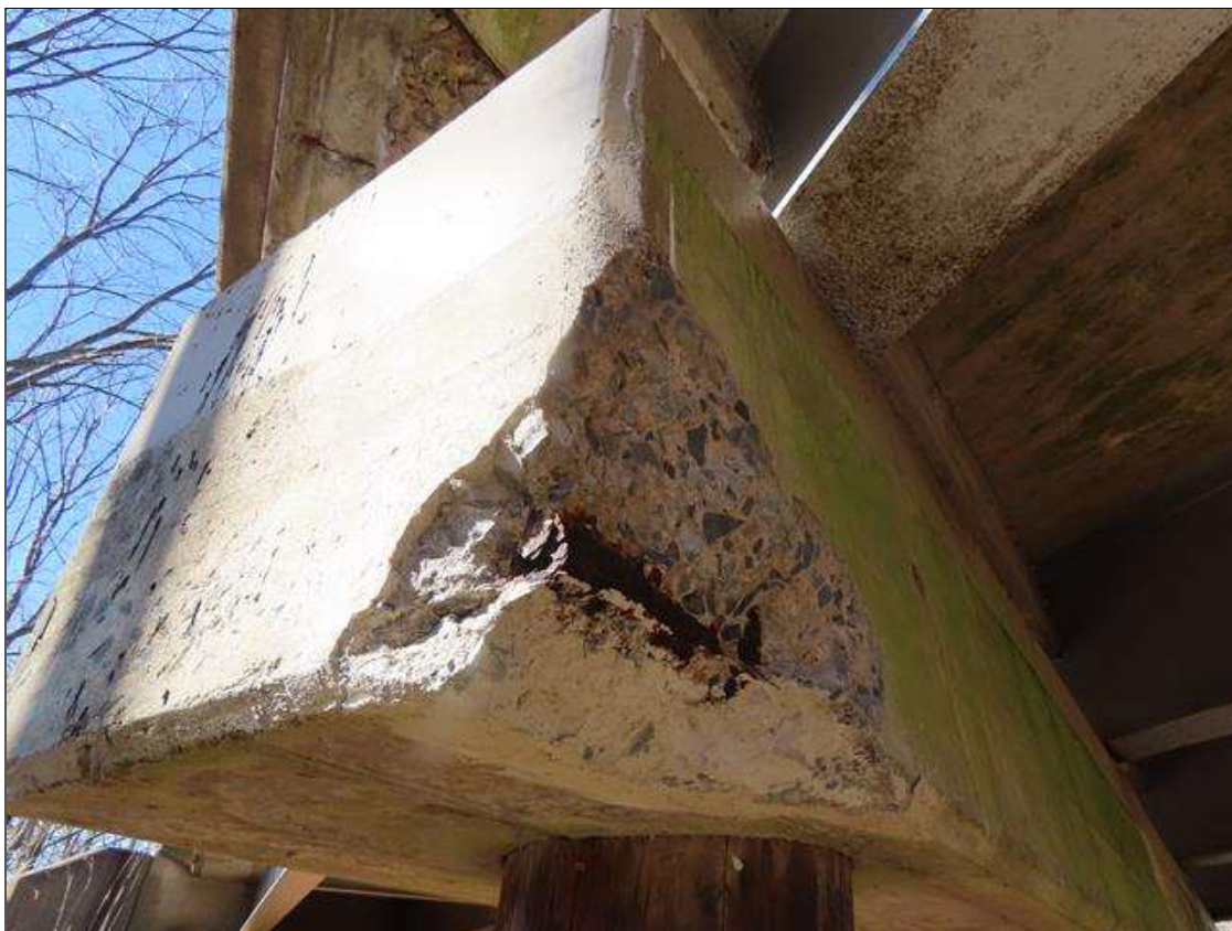
BENT 1 CAP - SPALLED PATCH (16IN L. X 12IN W. X 2.5IN D.) WITH EXPOSED & CORRODED (1/16IN SL) REBAR TO FAR RIGHT CORNER AT BOTTOM. (PAR)
