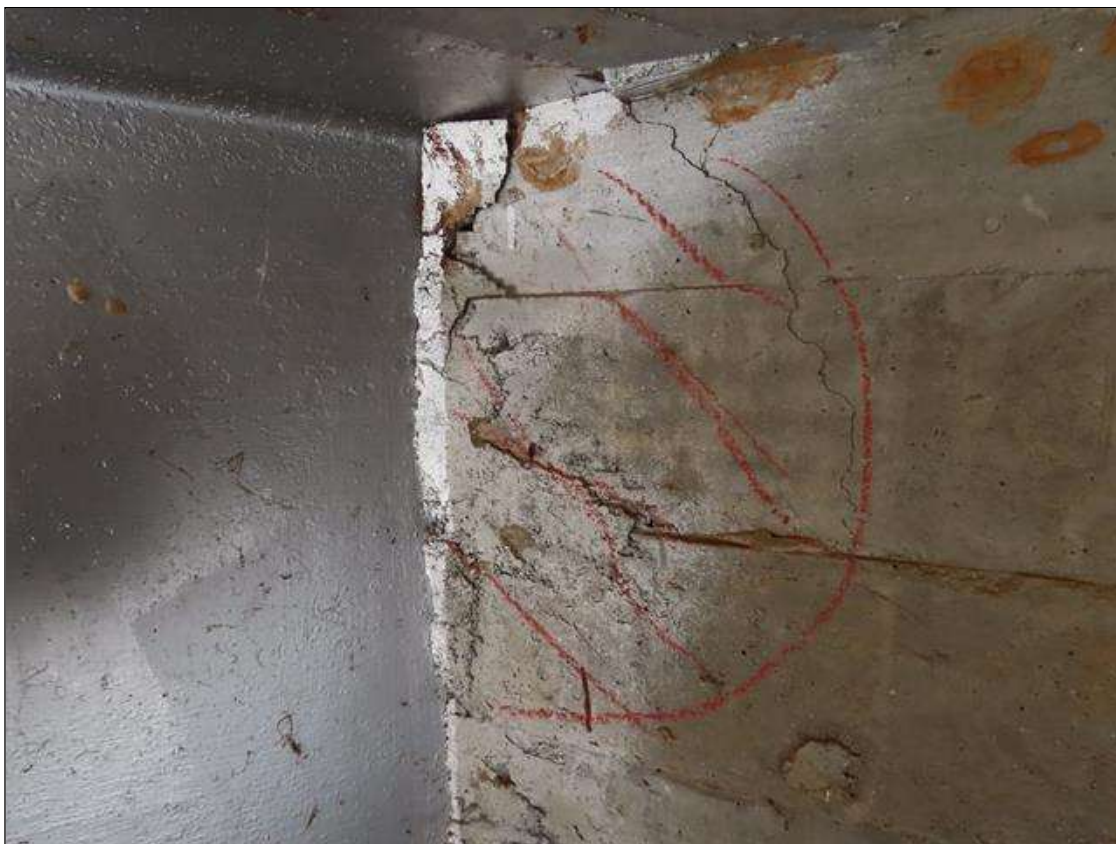
END BENT 2 ABUTMENT - DELAM (1SF) TO BACKWALL AT RIGHT SIDE OF BEAM 3
