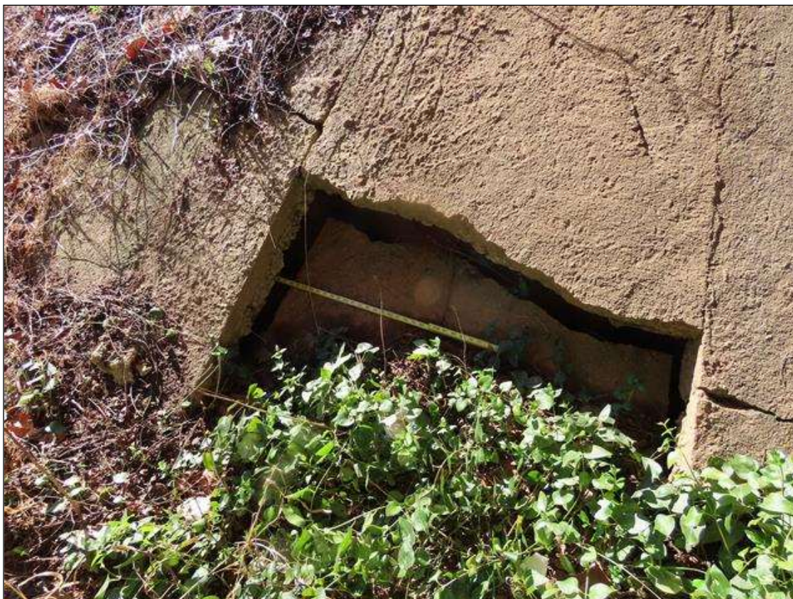
END BENT 1 SLOPE PROTECTION - SPALLED/BROKEN AREA (3FT L. X 3FT W.) WITH EROSION (UP TO 2FT D.) UNDER CONCRETE SLOPE PROTECTION AROUND BROKEN AREA, BELOW BAY 4. (PAR)
