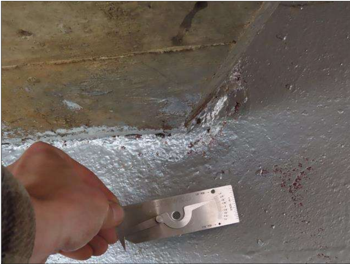
SPAN 4 BEAM 2 - ARRESTED WEB SECTION LOSS (UP TO 3/16IN SL, 5/16IN REMAIN) 5IN L. X 1.5IN W. AT FAR END DIAPHRAGM. (PAR)
