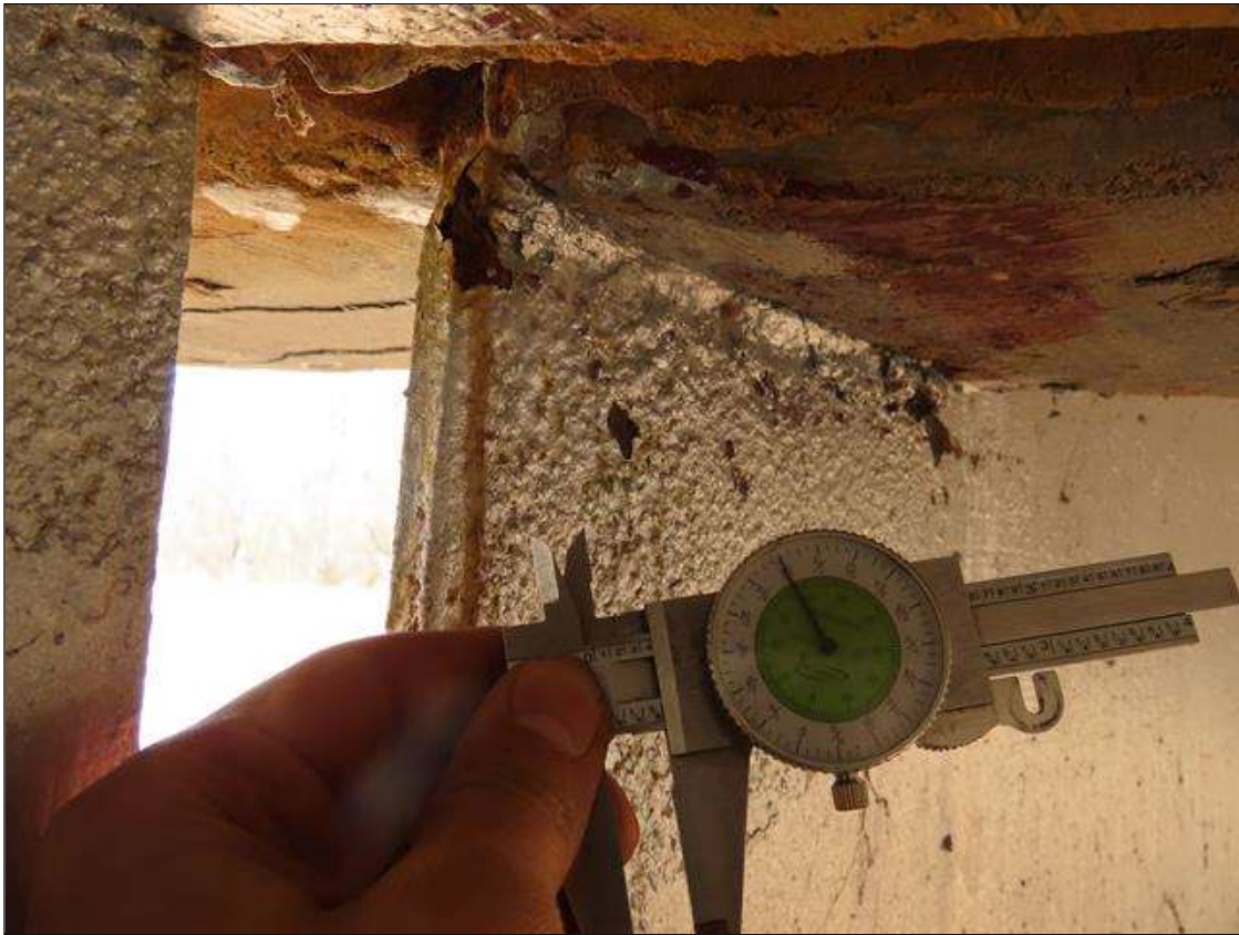
SPAN 4 BEAM 1 - PARTIALLY ARRESTED WEB SECTION LOSS (UP TO 1/8IN SL, 3/8IN REMAIN) 6IN L. X 1IN H. AT NEAR END DIAPHRAGM
