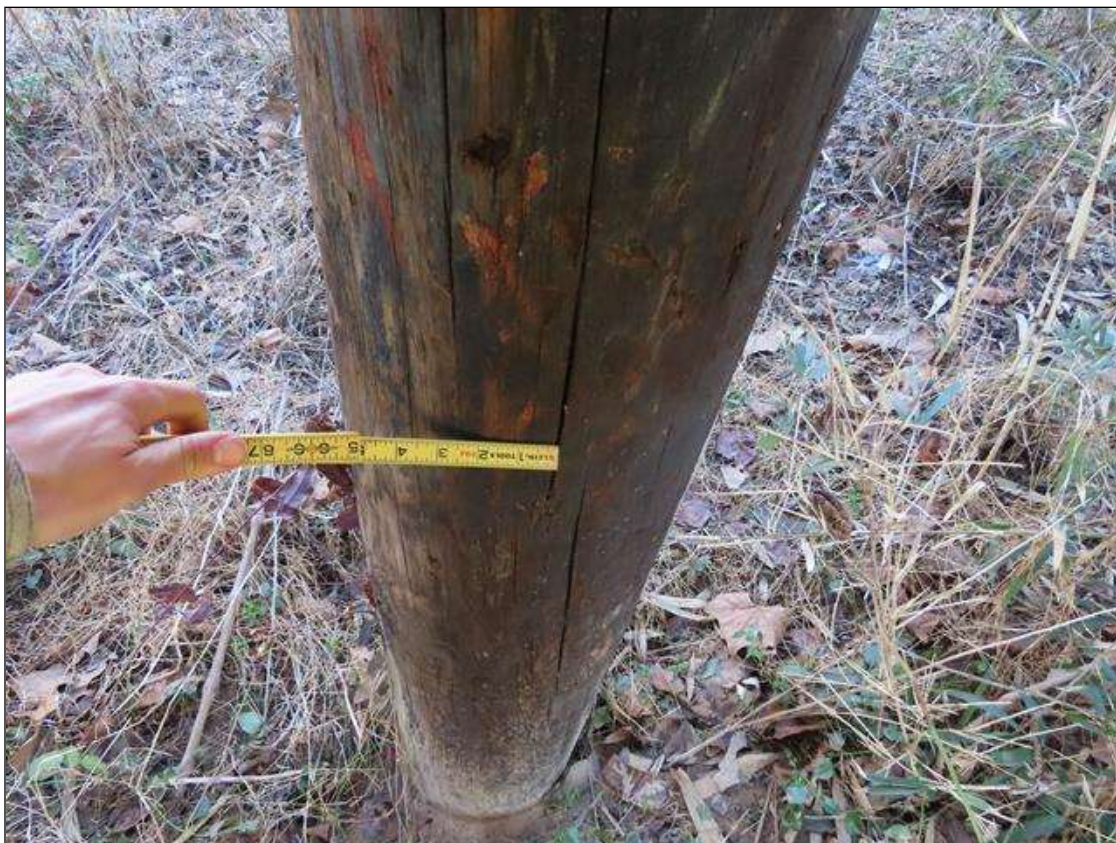
TYPICAL MINOR CHECKING THROUGHOUT PILES, BENT 1 PILE 1
