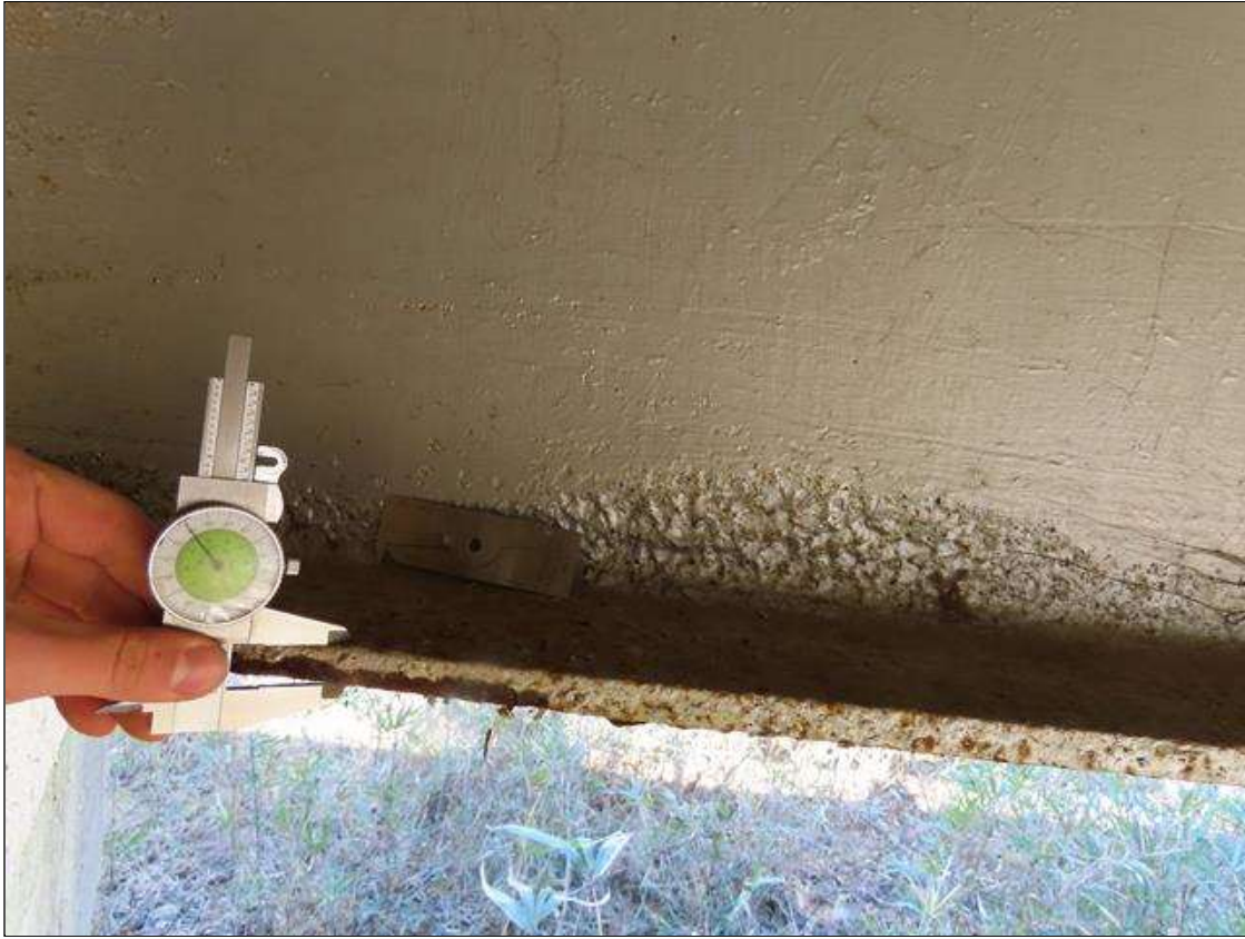
SPAN 2 BEAM 1 - BOTTOM FLANGE SECTION LOSS (UP TO 10%, 1/16IN SL, 9/16IN REMAIN) FULL W. FOR 2FT L. AT NEAR END, AND ARRESTED WEB SECTION LOSS (UP TO 3/16IN SL, 5/16IN REMAIN) 3FT L. X 3IN H. TO BOTTOM AT NEAR END. (PAR)
