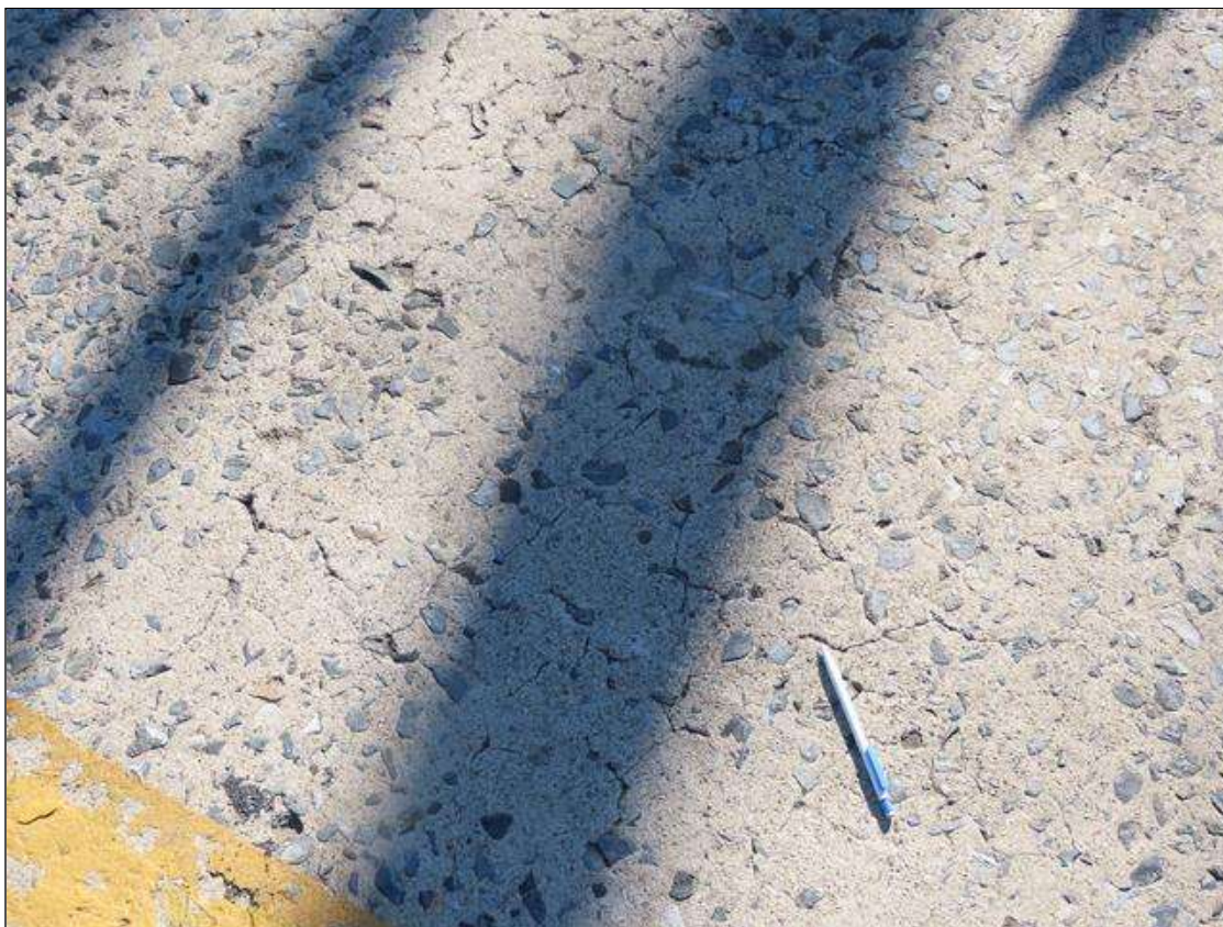
TYPICAL 1/32IN MAP CRACKING & MODERATE TO HEAVY WEAR WITH EXPOSED AGGREGATE THROUGHOUT SPAN 1 RIGHT LANE
