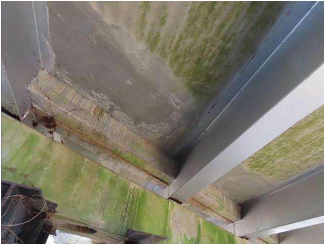
TYPICAL SOUND PATCHING (UP TO 5FT L. X 2FT W.) TO DECK ADJACENT TO BENT 2, SPAN 2 BAY 1 & 2 AT FAR END.
