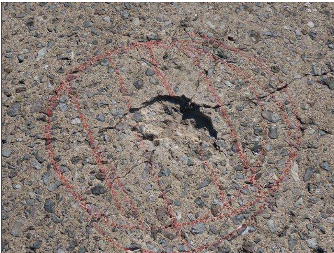
SPAN 5 DECK - SPALL/DELAM (2SF X 1/2IN D.) WITH EXPOSED REBAR IN LEFT LANE 18IN FROM NEAR END. (PAR)
