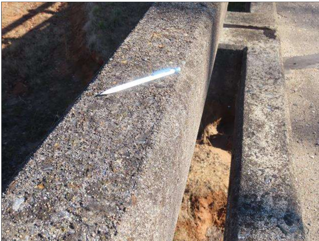
TYPICAL MINOR TO MODERATE WEAR WITH EXPOSED AGGREGATE THROUGHOUT RAILS, SPAN 3 LEFT SIDE
