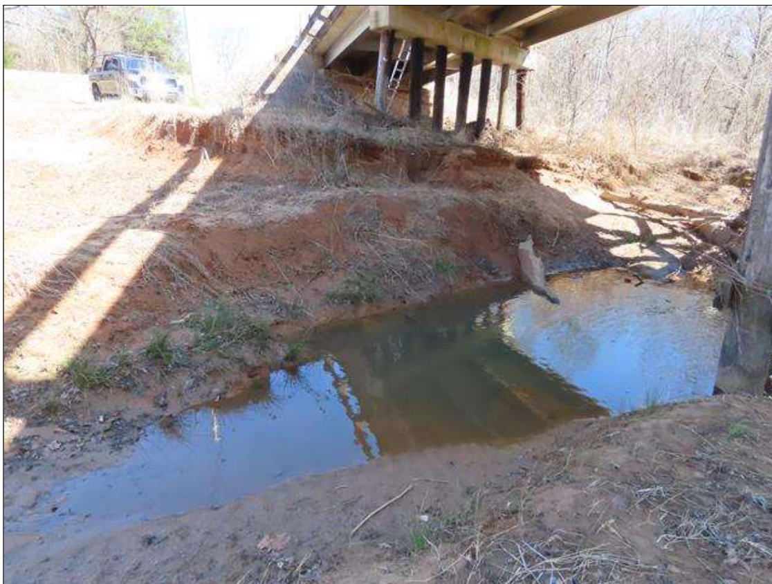
STREAM BANK BELOW SPAN 4 - BANK EROSION (UP TO 6FT H. X 20FT W. X 50FT L.) AT FAR SIDE OF BENT 3
