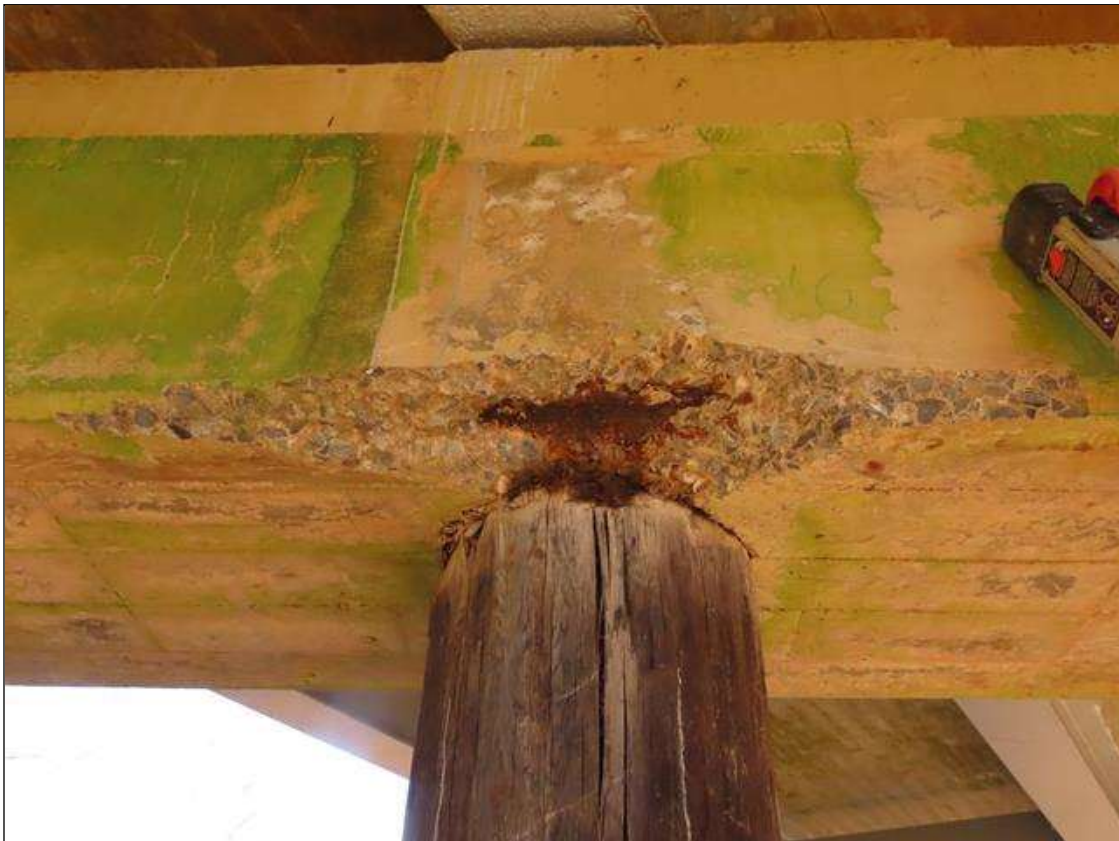
BENT 1 CAP - SPALL (30IN L. X 8IN W. X 2.5IN D.) WITH EXPOSED & CORRODED (1/16IN SL) REBAR TO NEAR SIDE OVER PILE 3. (PAR)
