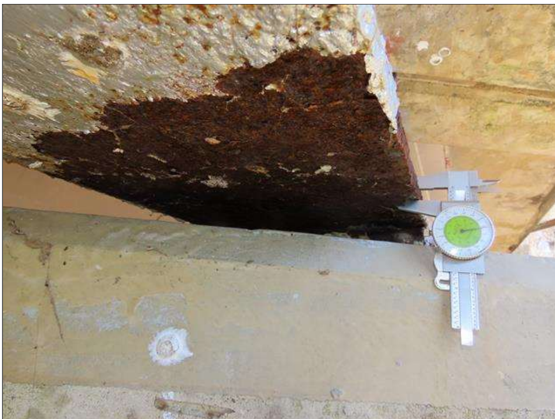
SPAN 3 BEAM 4 - TAPERED BOTTOM FLANGE SECTION LOSS (UP TO 20%, 1/4IN SL, 3/8IN REMAIN AT EDGE) FULL W. FOR 12IN L. AT FAR END
