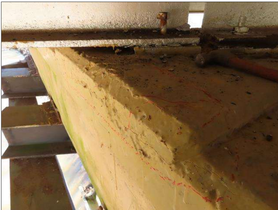
BENT 2 CAP - DELAM (2FT L. X 6IN W.) TO FAR SIDE AT TOP EDGE BELOW BEAM 3. (DOES NOT EXTEND BELOW BEARING)
