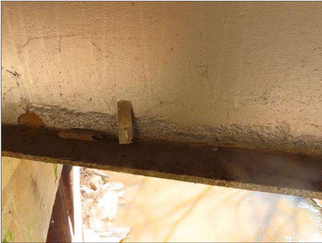
SPAN 3 BEAM 3 - ARRESTED WEB SECTION LOSS (UP TO 1/8IN SL, 3/8IN REMAIN) 2.5IN H. X 2.5FT L. TO BOTTOM AT NEAR END OF REPAIR
