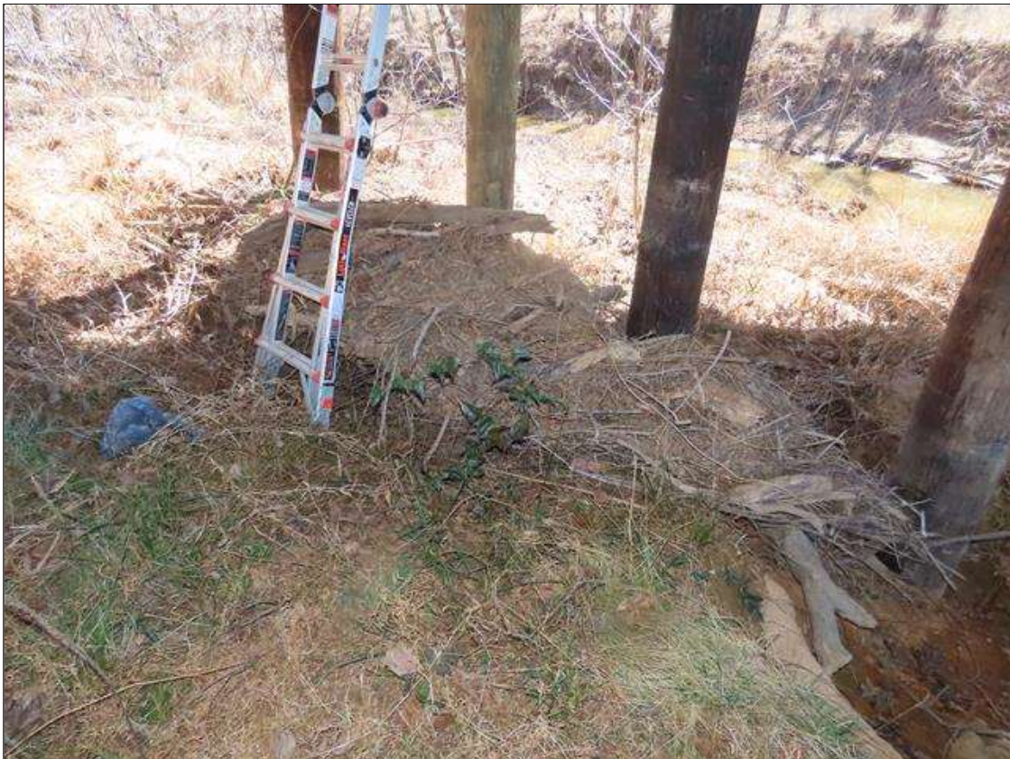
DRIFT (25CUFT) AT FAR SIDE OF BENT 4 AT PILES 4-7
