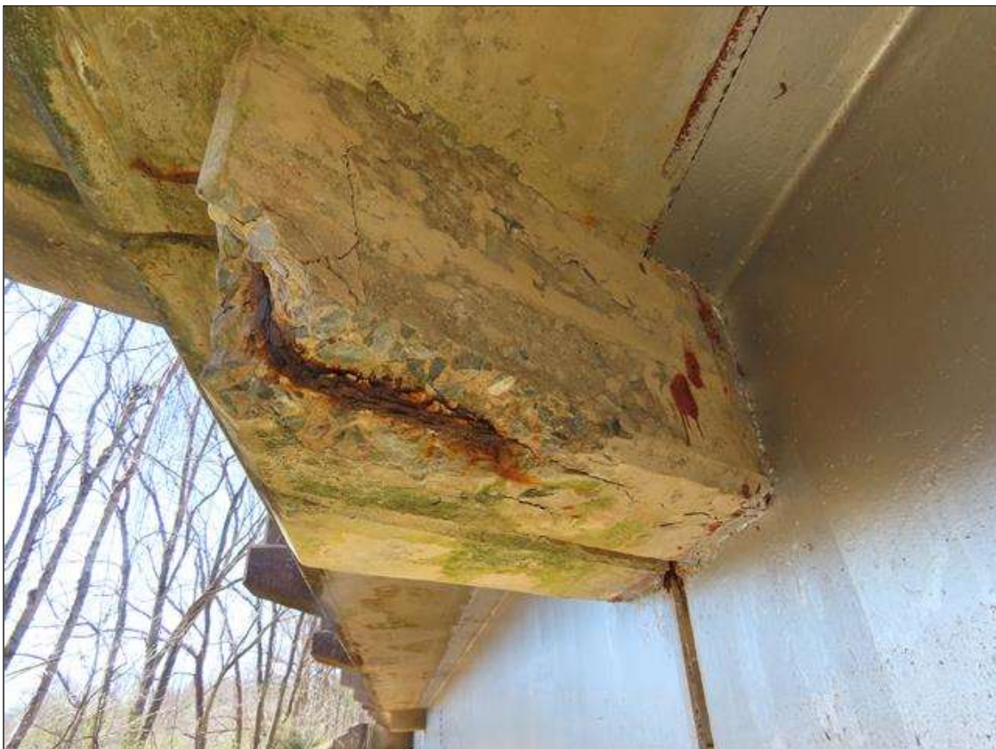
SPAN 3 BEAM 4, NEAR END DIAPHRAGM - SPALL (16IN L. X 8IN W. X 2IN D.) WITH EXPOSED & CORRODED REBAR (1/16IN SL) AT RIGHT SIDE OF BEAM. (PAR)
