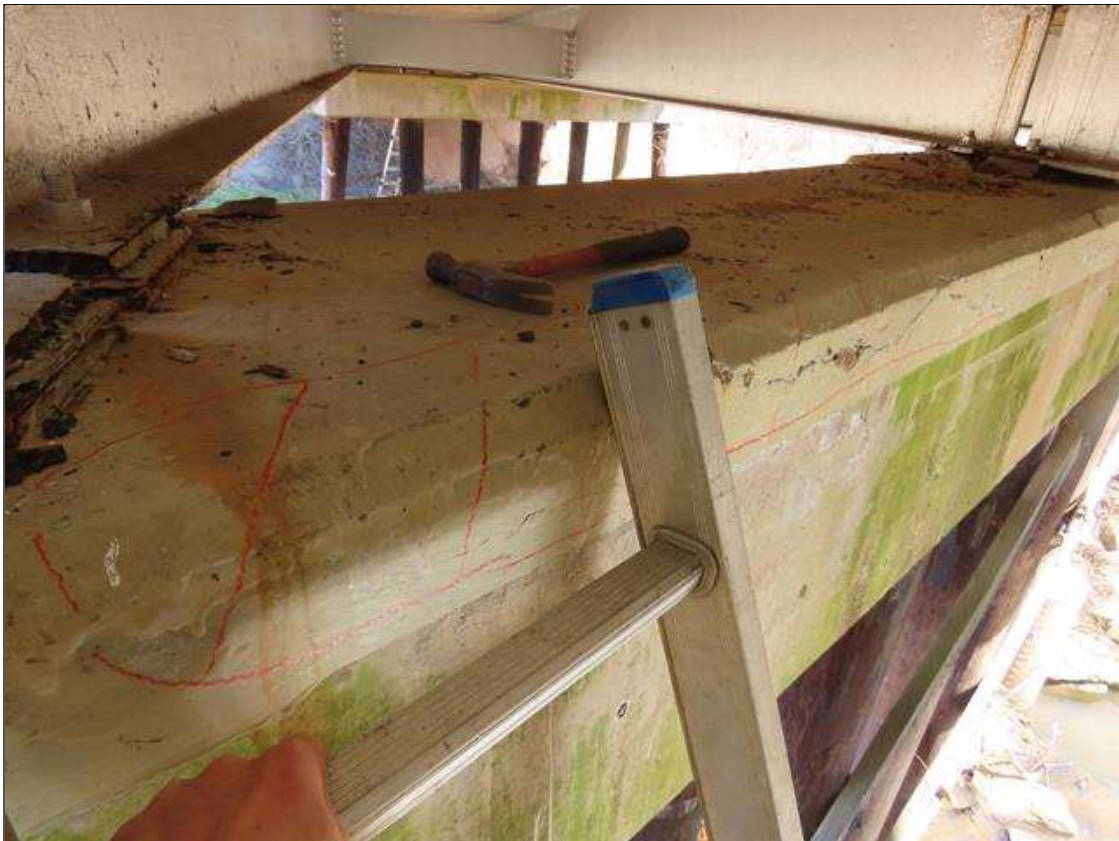
BENT 3 CAP - DELAM (10FT L. X 8IN W.) TO NEAR SIDE TOP EDGE STARTING IN BAY 1. (DOES NOT EXTEND BELOW BEARINGS)
