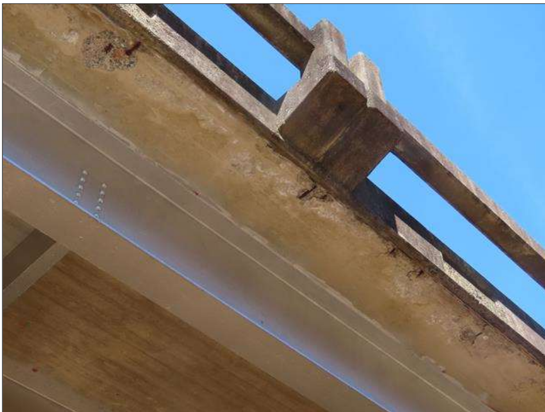
SPAN 4 DECK - X5 SPALLS/DELAM (UP TO 1SF X 1IN D.) WITH EXPOSED & SCALING REBAR TO BOTTOM OF RIGHT SIDE OVERHANG AT MID-SPAN
