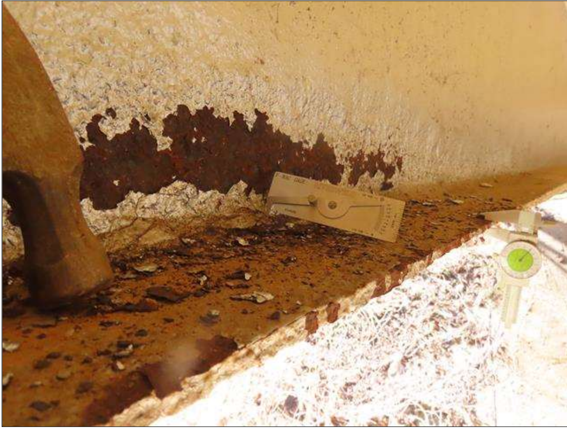
SPAN 1 BEAM 4 - TAPPERED BOTTOM FLANGE SECTION LOSS (UP TO 25%, 3/8IN SL, 1/4IN REMAIN) 8IN W. FOR 8FT L., AND WEB SECTION LOSS (UP TO 1/4IN SL, 1/4IN REMAIN) UP TO 10IN H. FOR 8FT L. AT FAR END. (PAR)
