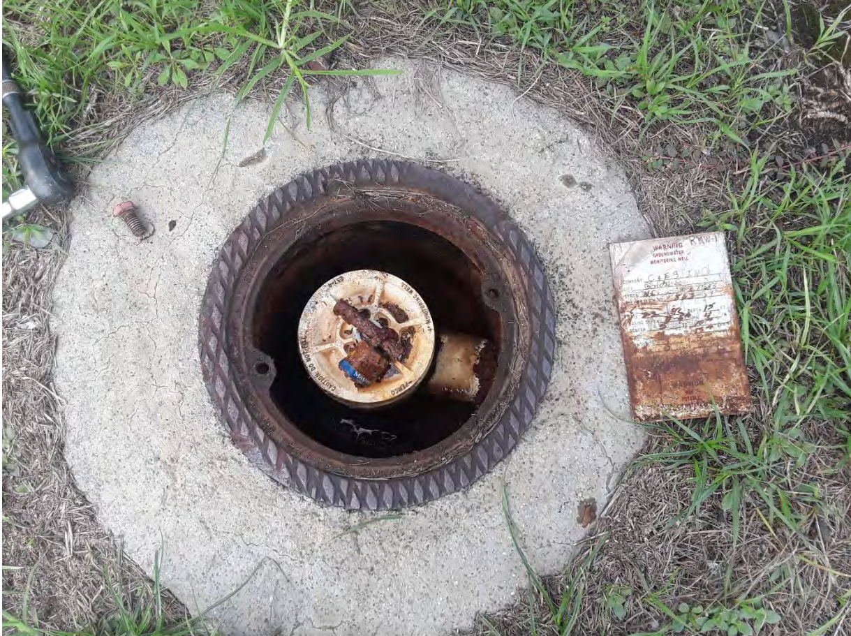
Photo 3 – A close-up view of well RMW-1 (not abandoned) – note horizontal pipe connected to well.
