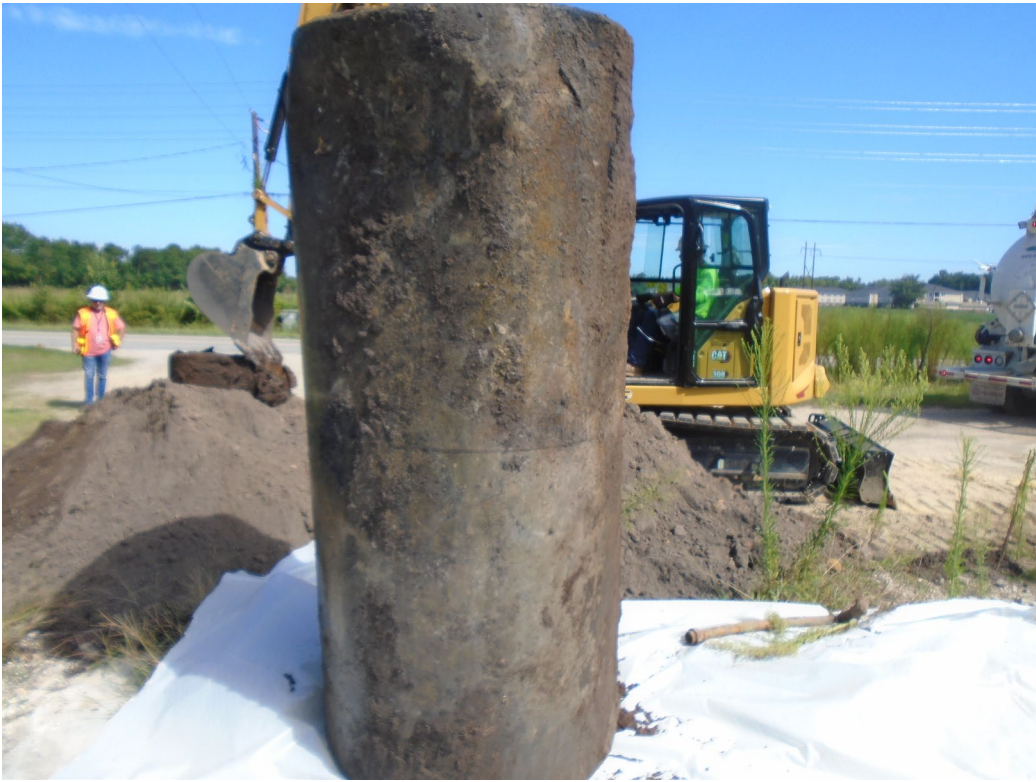
Photograph 5 – The 1,000-gallon capacity UST being positioned so the bottom can be inspected for holes.
