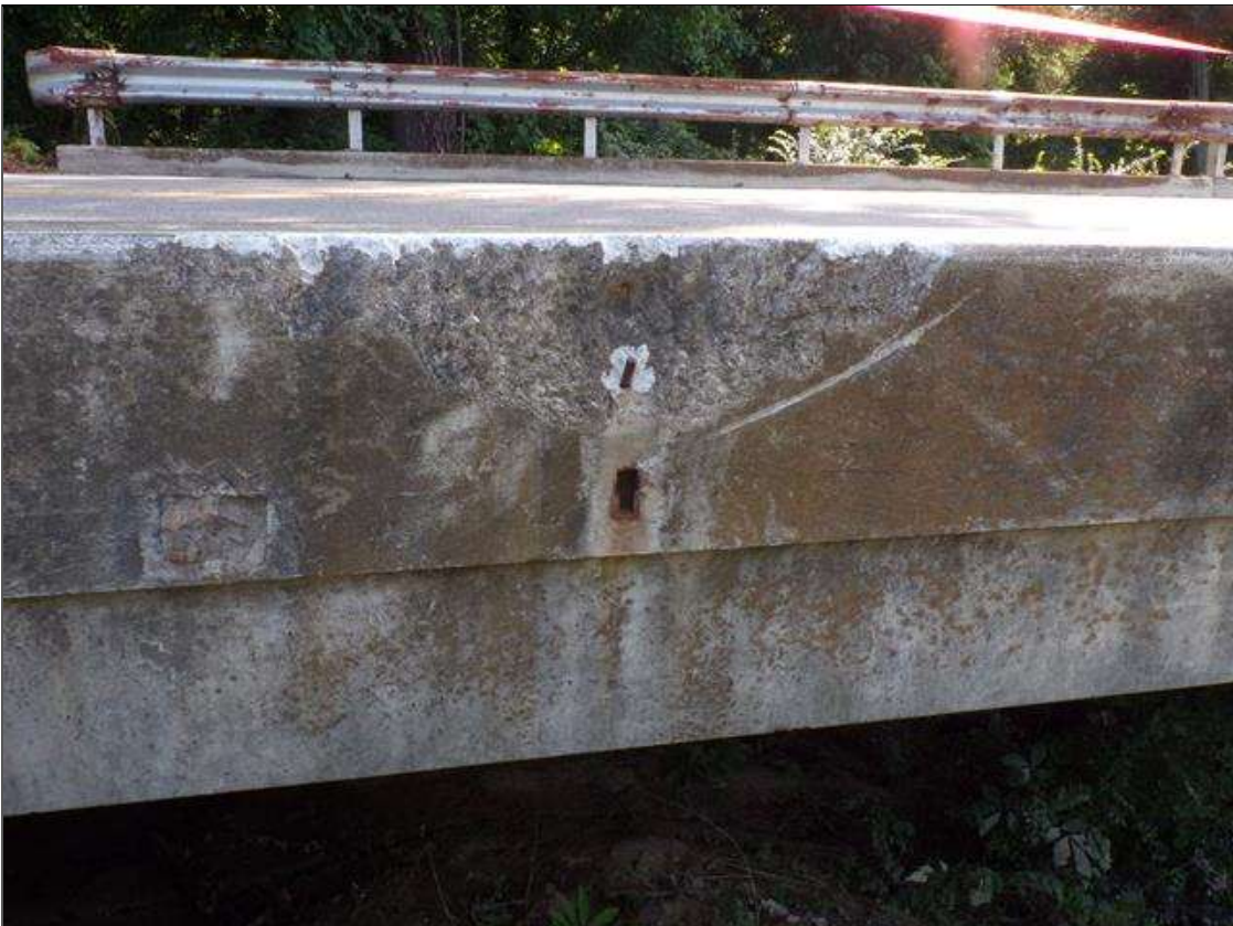
Span 4 Left Bridge Rail: PAR-Left rail in span 4 has impact damage and has completely separated from structure along length. All post are missing with spalling up to 1 foot wide x 4 inches deep at post connections to curbing.
