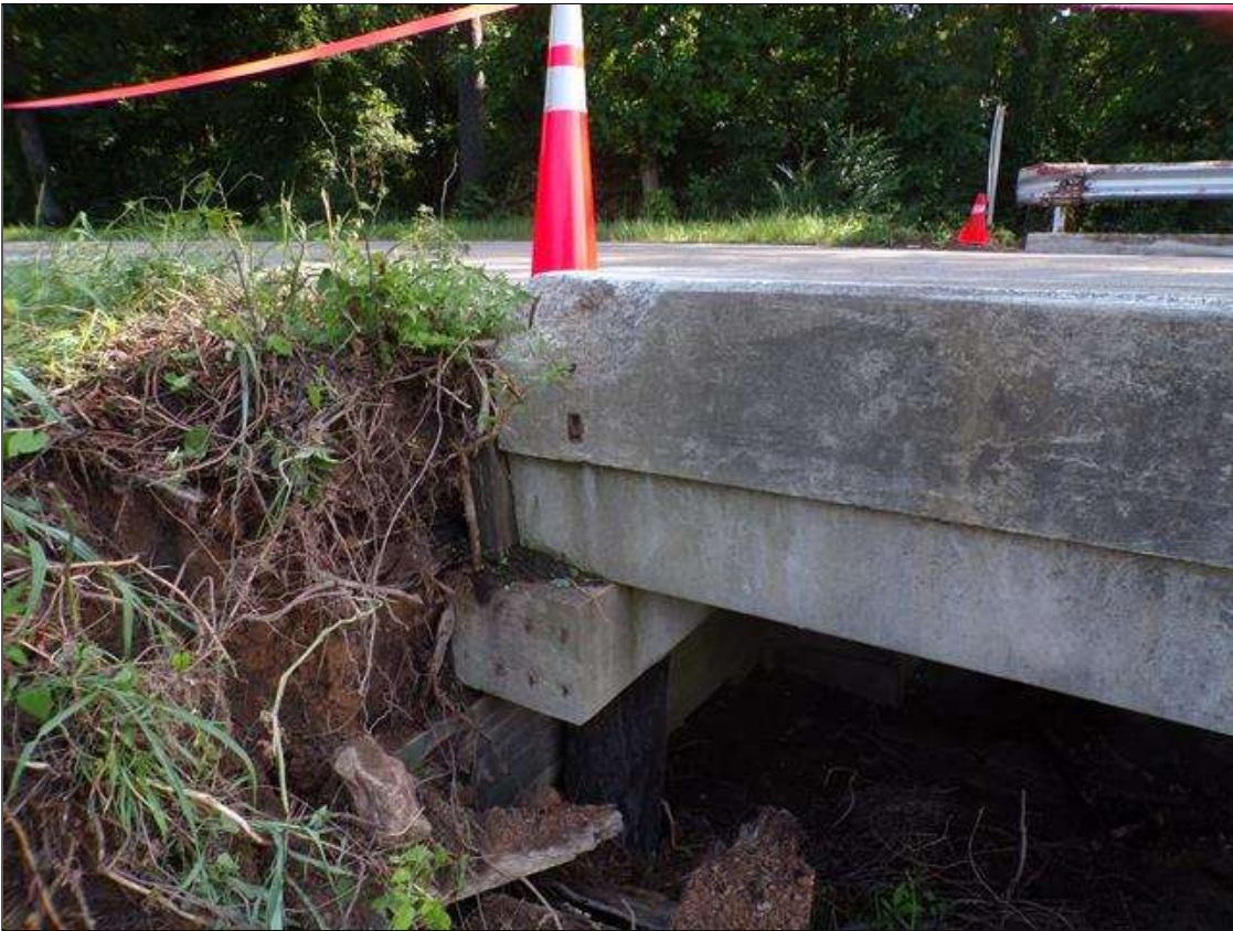
Span 4 Left Bridge Rail: PAR-Left rail in span 4 has impact damage and has completely separated from structure along length. All post are missing with spalling up to 1 foot wide x 4 inches deep at post connections to curbing.
