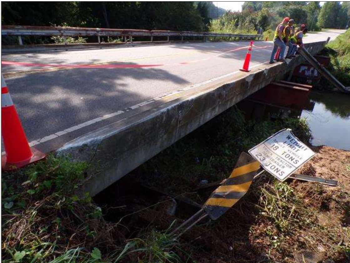
Span 4 Left Bridge Rail: PAR-Left rail in span 4 has impact damage and has completely separated from structure along length. All post are missing with spalling up to 1 foot wide x 4 inches deep at post connections to curbing.
