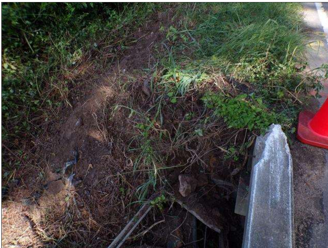
End Bent 2 Abutment: PAR- End Bent 2 bulkhead is broken and missing in a 5 foot long area at left end due to impact damage.
