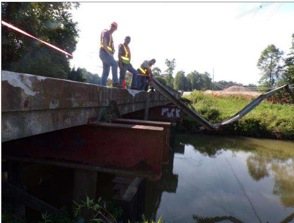
Span 3 Left Bridge Rail: PAR-Left rail in span 3 has impact damage and has completely separated from structure from midspan to bent 3. All post are missing in this area with spalling up to 1foot wide x 4 inches deep at post connections to curbing.
