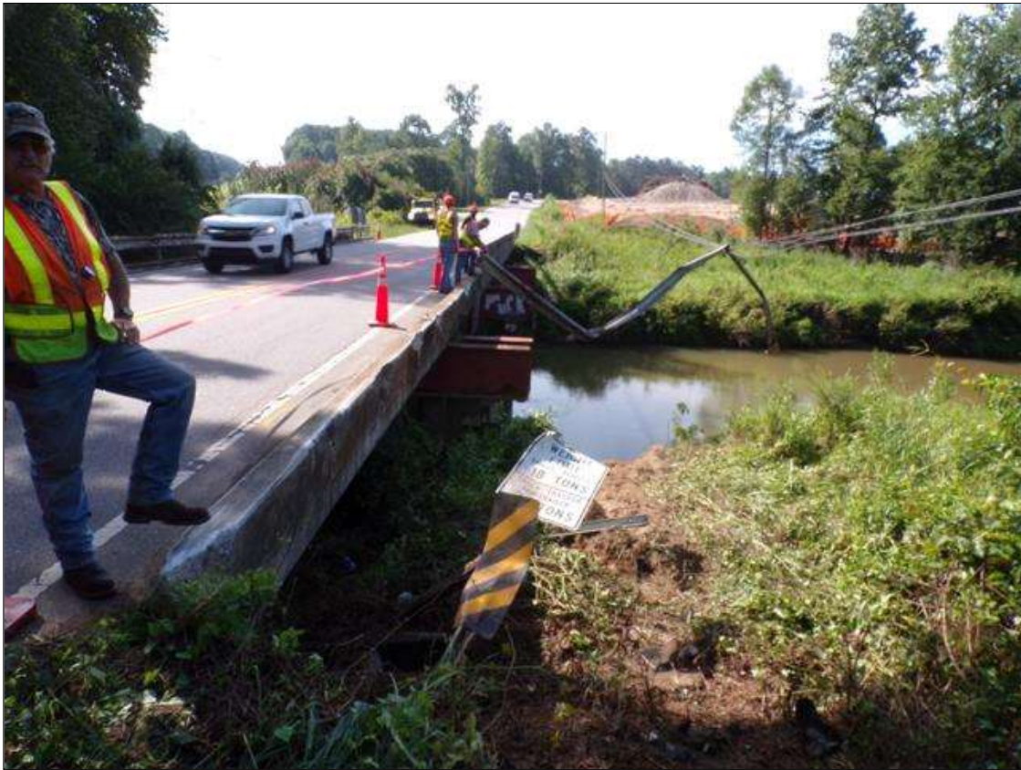
Span 4 Left Bridge Rail: PAR-Left rail in span 4 has impact damage and has completely separated from structure along length. All post are missing with spalling up to 1 foot wide x 4 inches deep at post connections to curbing.
