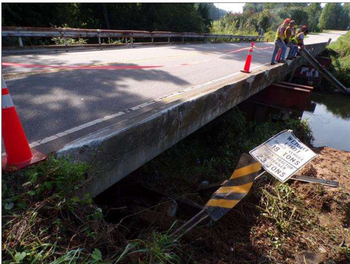
PAR-Posting sign SV 18 TTST 23 and Delineator missing from right shoulder at north approach.
