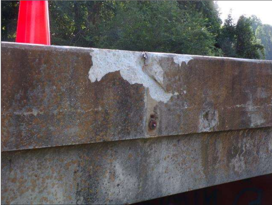
Span 3 Left Bridge Rail: PAR-Left rail in span 3 has impact damage and has completely separated from structure from midspan to bent 3. All post are missing in this area with spalling up to 1foot wide x 4 inches deep at post connections to curbing.
