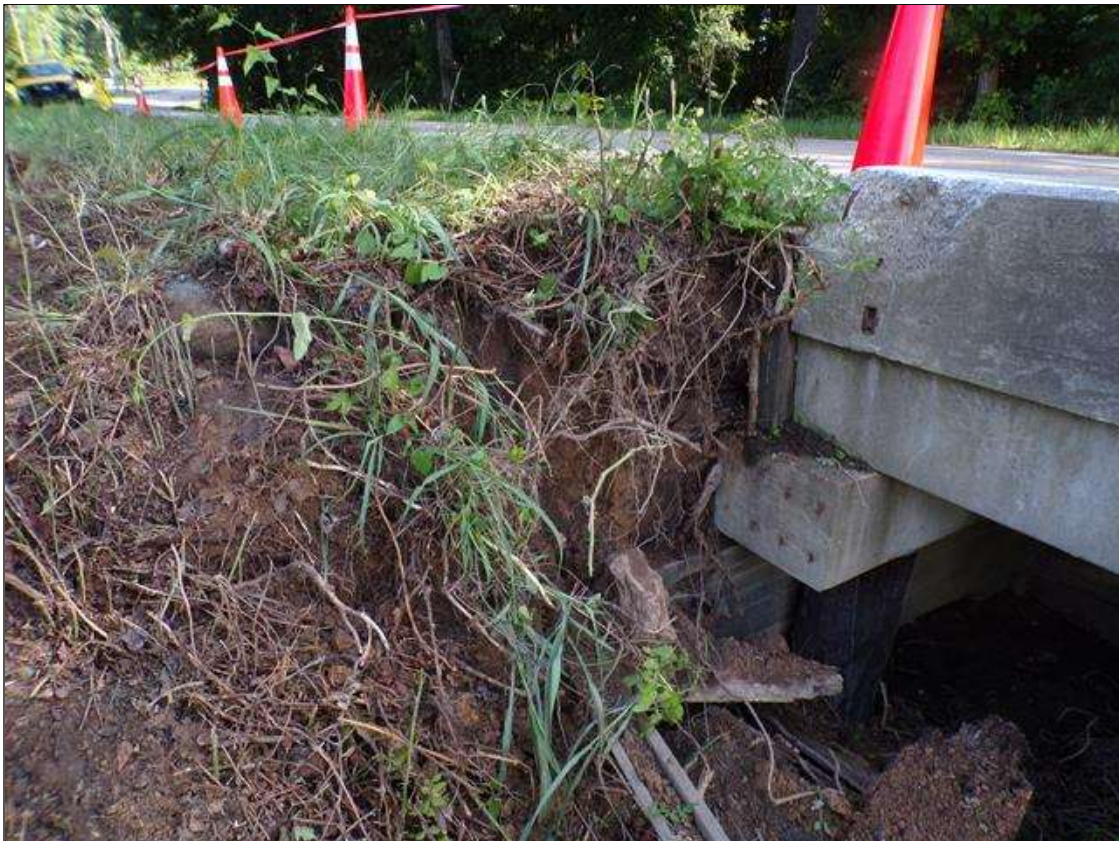
End Bent 2 Abutment: PAR- End Bent 2 bulkhead is broken and missing in a 5 foot long area at left end due to impact damage.
