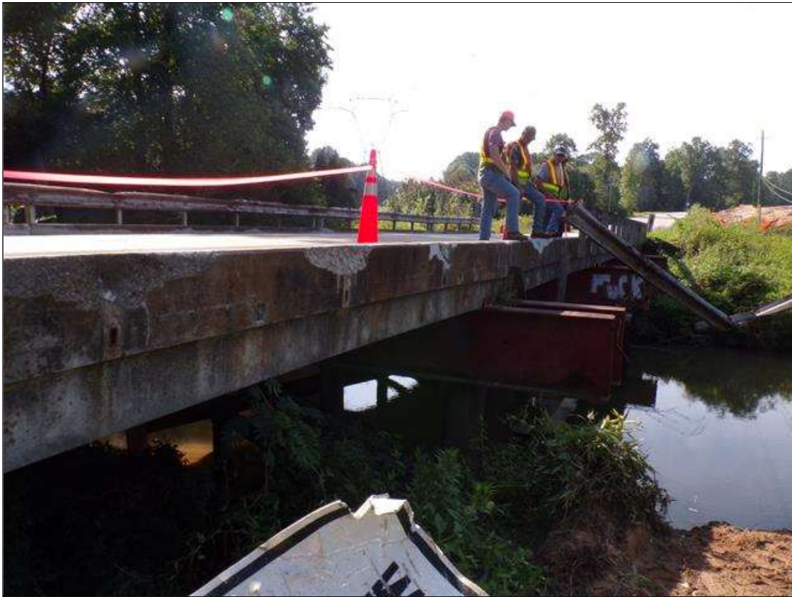
Span 4 Left Bridge Rail: PAR-Left rail in span 4 has impact damage and has completely separated from structure along length. All post are missing with spalling up to 1 foot wide x 4 inches deep at post connections to curbing.
