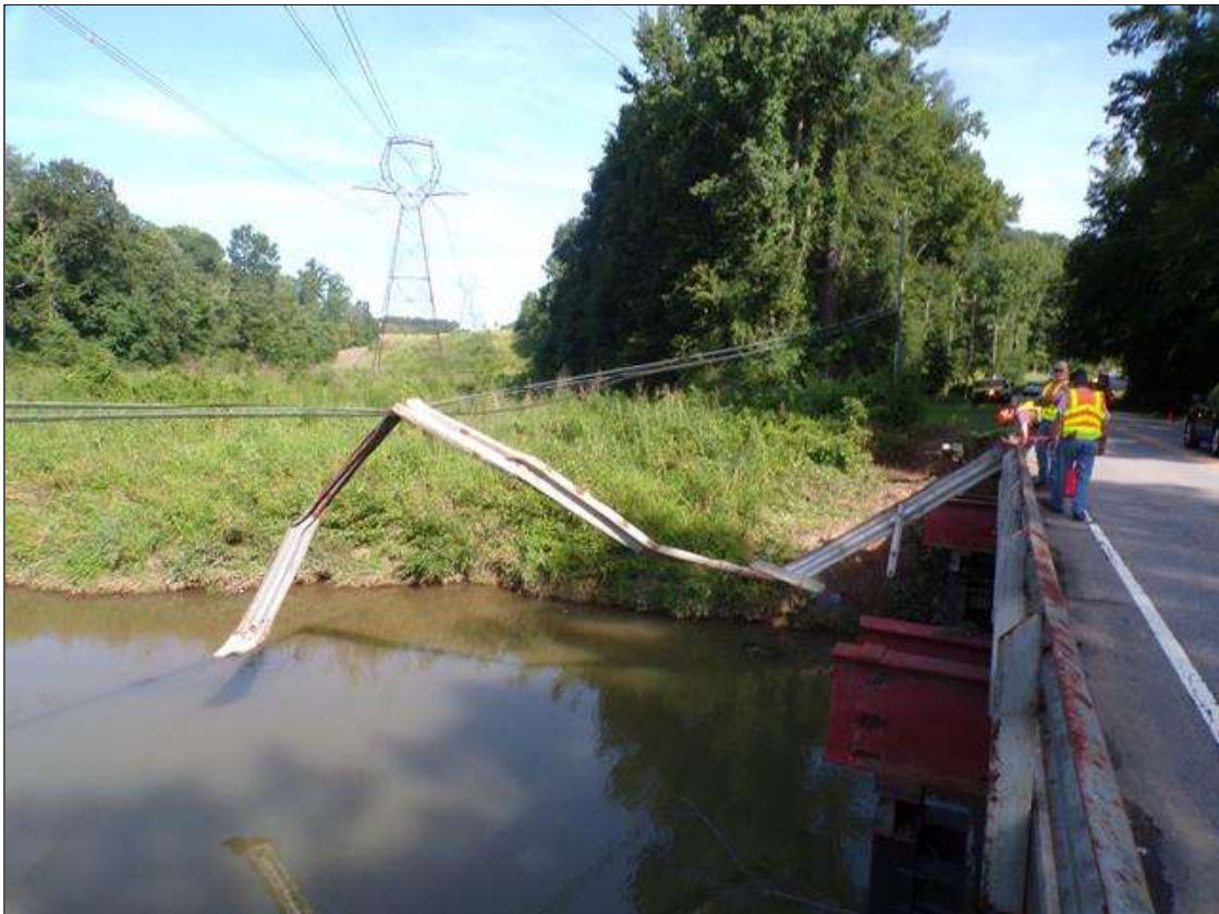
Span 4 Left Bridge Rail: PAR-Left rail in span 4 has impact damage and has completely separated from structure along length. All post are missing with spalling up to 1 foot wide x 4 inches deep at post connections to curbing.
