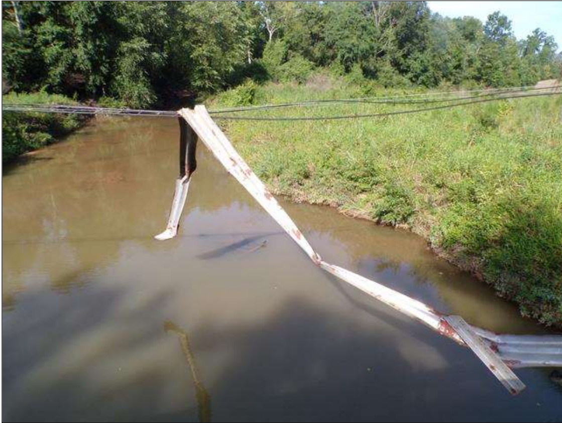
Span 4 Left Bridge Rail: PAR-Left rail in span 4 has impact damage and has completely separated from structure along length. All post are missing with spalling up to 1 foot wide x 4 inches deep at post connections to curbing.
