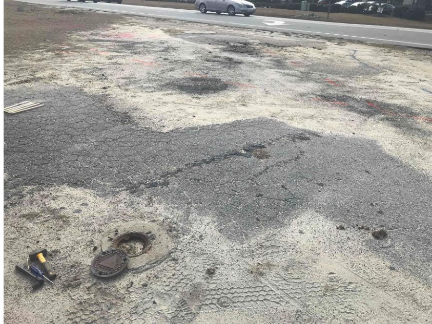
Photo #5 View of the on-site abandoned monitoring well identified during the geophysical investigation; facing south.
