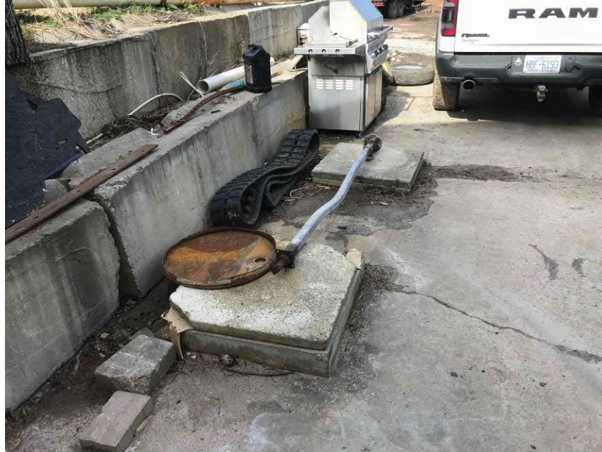
Photo #5 View of the on-site septic tank located north of the on-site building; facing northwest.
