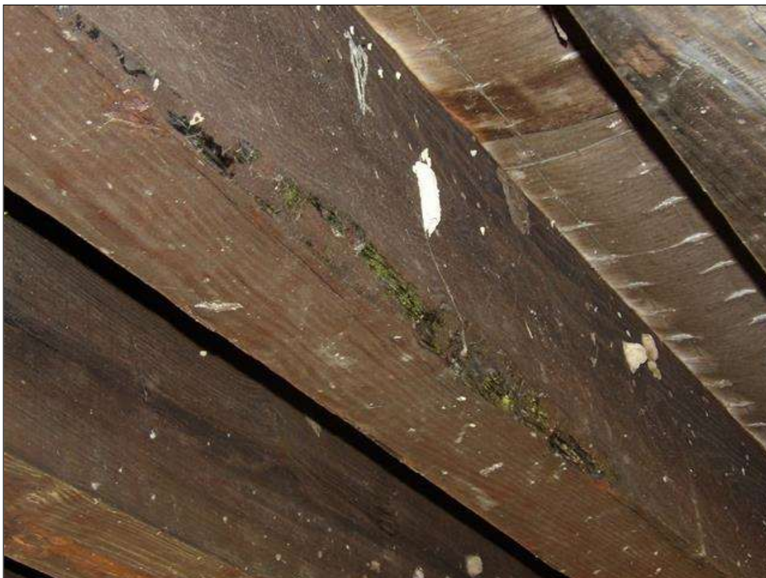
Span 1 Beam 5: SHAKE 30 INCHES LONG. X 2 INCHES WIDE X 1 INCH DEEP TO BOTTOM EAST FACE AT MID-SPAN
