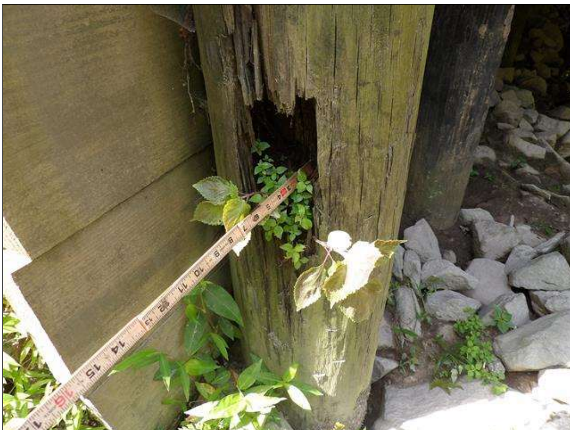
End Bent 1 Abutment: PAR--EAST SIDE ABUTMENT SUPPORT PILE - DECAY 12 INCHES HEIGHT. X 4 INCHES WIDE X 4 INCHES DEEP TO RIGHT SIDE, 2 FEET FROM BOTTOM.
