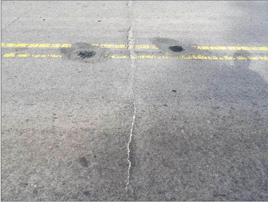
Span 1 Wearing Surface: ASPHALT WEARING SURFACE OVER END BENT 1 - TRANSVERSE CRACKING UP TO 1 INCH X FULL WIDE. THROUGHOUT, AND ASPHALT WEARING SURFACE OVER BENT 1 & CRUTCH BENTS - TRANSVERSE CRACKING UP TO 1/2 INCHES X FULL WIDTH WITH BROKEN ASPHALT WEARING SURFACE NEAR CENTER LINE 2.5 FEET WIDE X 3 INCHES LONG. BENT 1 SHOWN
