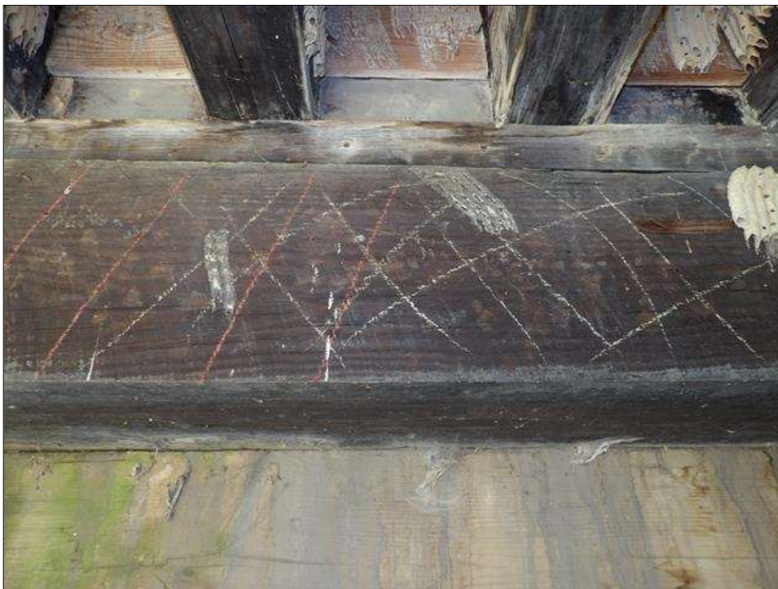
End Bent 1 Cap 1: PAR--HOLLOW WHEN SOUNDED 6 FEET LONG. X FULL HEIGHT STARTING OVER COLUMN 3.
