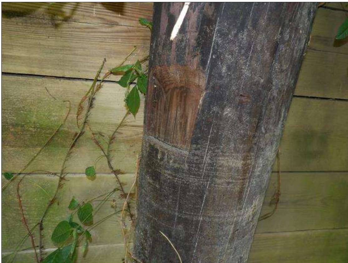
End Bent 2 Pile 1: SECTION LOSS 6 INCHES X 6 INCHES X 1 INCH TO WEST FACE, 2 FEET FROM TOP
