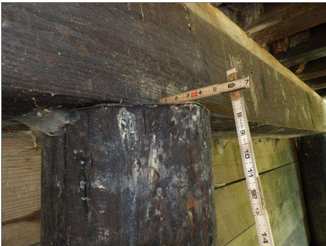
End Bent 1 Pile 2: PAR--BEARING LOSS UP TO 3 INCHES AT TOP OF PILE DUE TO PILE OUT OF PLUM.
