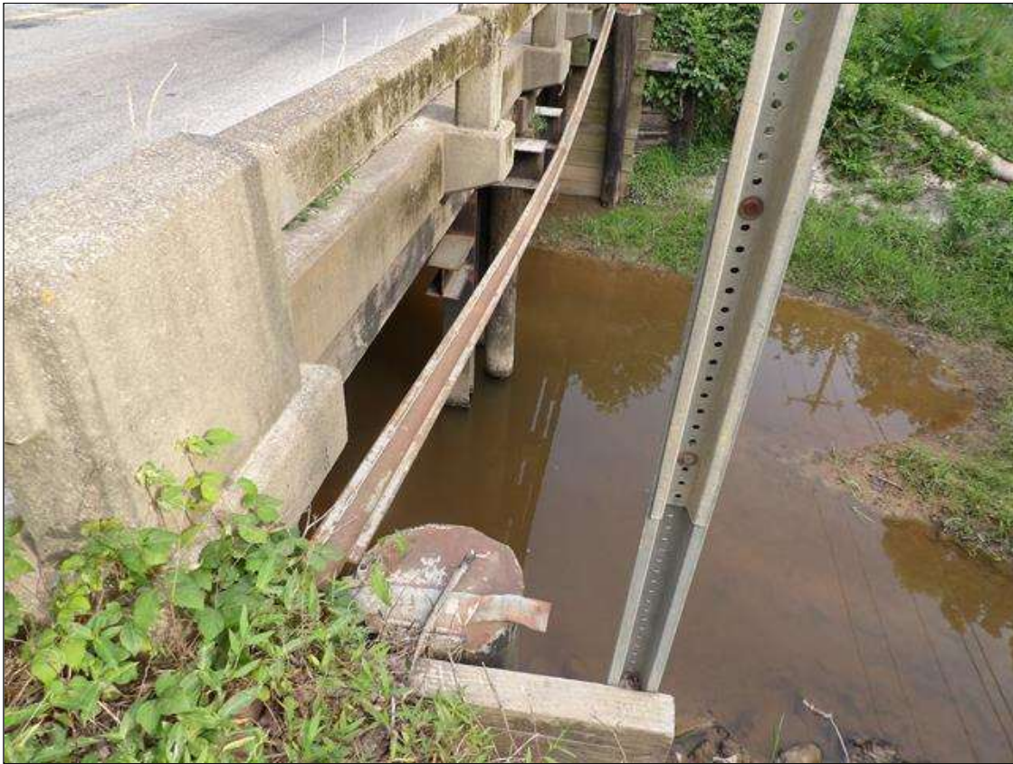
Abandoned/sagging utility pipe right side of bridge
