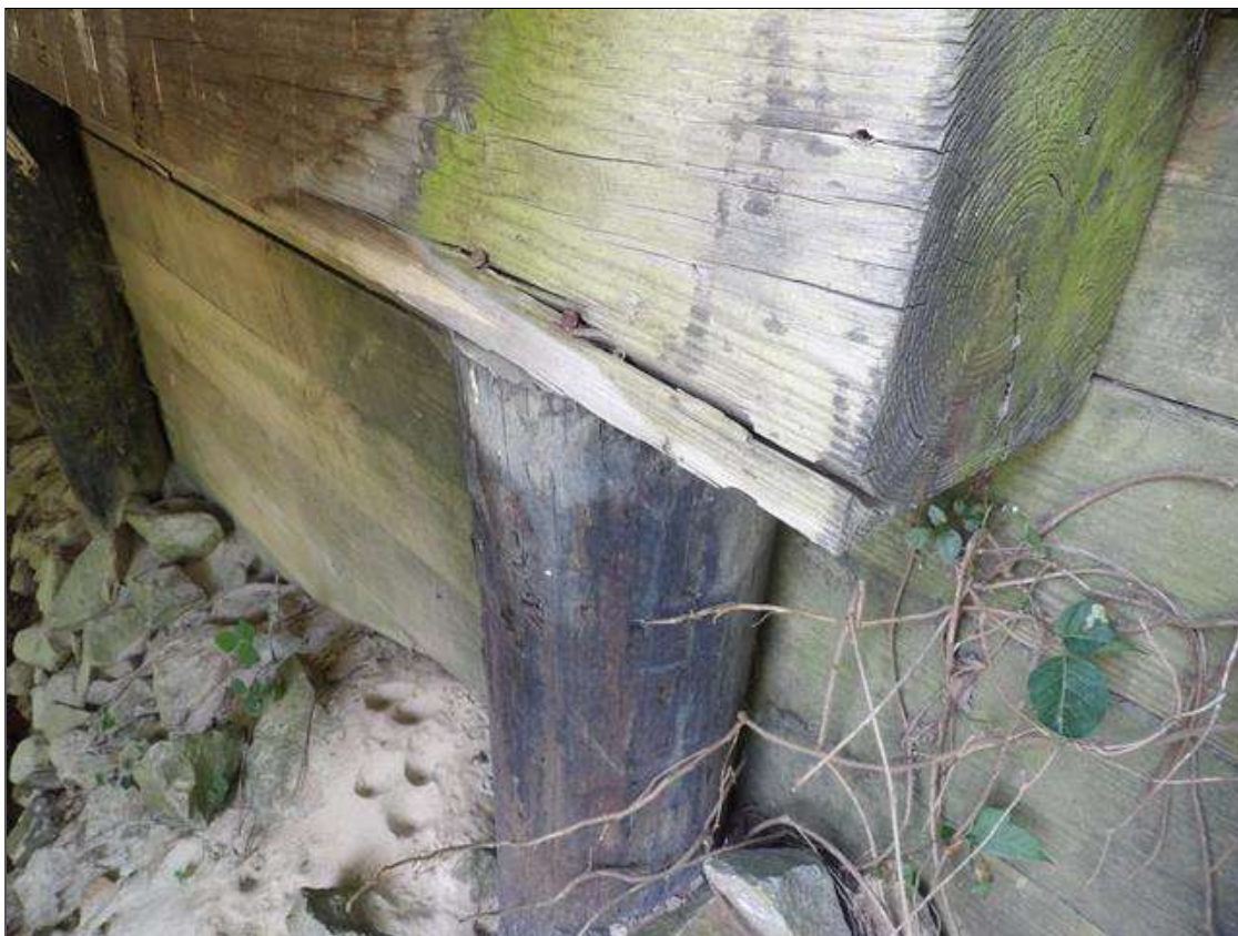
End Bent 1 Cap 1: SPLIT 24 INCHES LONG X 2 INCHES X 2 INCHES TO BOTTOM LEFT OVER PILE 1 AT NAIL LOCATION
