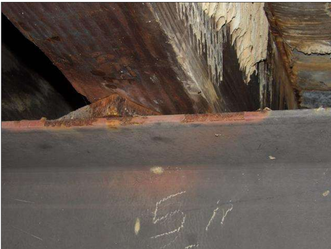
Span 2 Beam 4: NEAR BEARING AT CRUTCH BENT - SHIM PLATE SLIGHTLY SHIFTED
