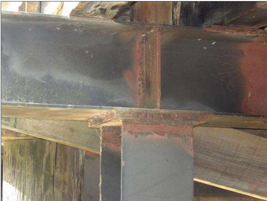
Typical surface corrosion on crutch bents
