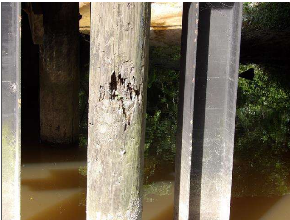
Bent 1 Pile 4: 10" X 8" X 1 1/2" DEEP AREA OF DECAY WEST FACE MID HEIGHT
