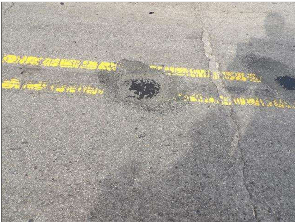
Span 1 Wearing Surface: SOUND PATCH, 1 FOOT X 1 FOOT AT FAR END, CENTER OF ROADWAY
