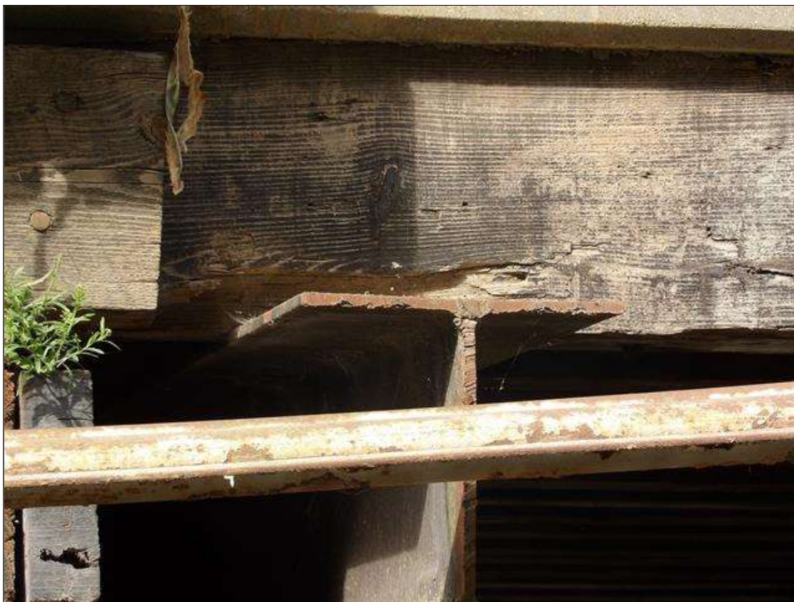
Span 2 Beam 19: SECTION LOSS 21 INCHES LONG. X 2 INCHES DEEP X 2 INCHES WIDE TO BOTTOM WEST FACE AT NEAR END
