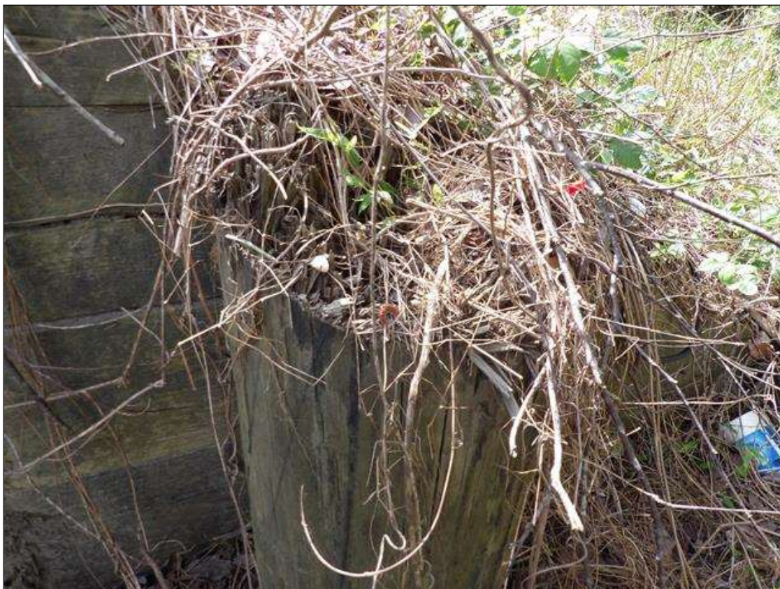
PAR--Southwest wingwall top 1' deep x full circumference area of decay to top holdback pile with 40% average remaining
