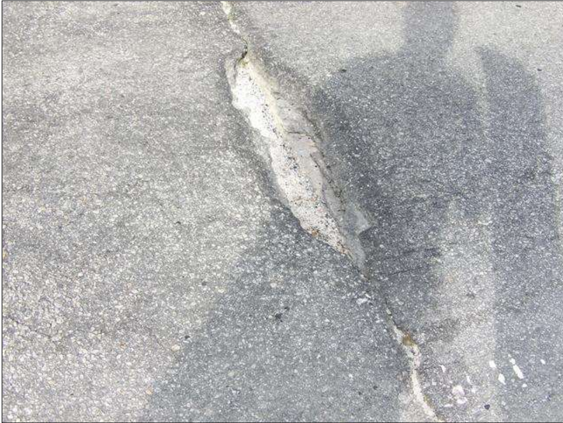
Span 1 Wearing Surface: PAR--SPALL/POTHOLE OVER ABUTMENT 1 2 FEET LONG. X 8 INCHES WIDE. X 3 INCHES DEEP NORTHBOUND TRAVEL LANE STARTING 2 FEET FROM RIGHT SHOULDER.
