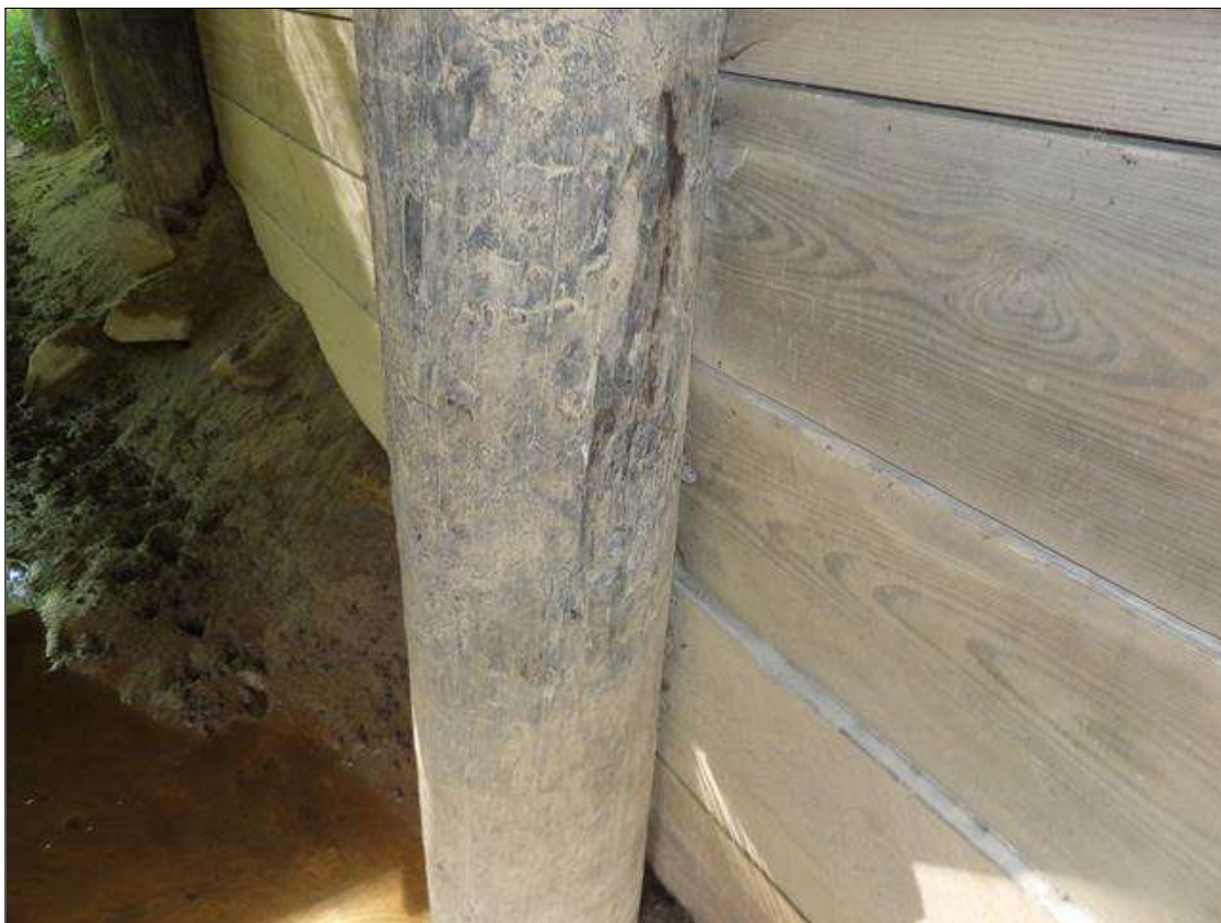
End Bent 2 Pile 3: DECAY 16 INCHES HEIGHT. X 6 INCHES WIDE X 1/2 INCHES DEEP TO EAST FACE, 2 FEET FROM BOTTOM
