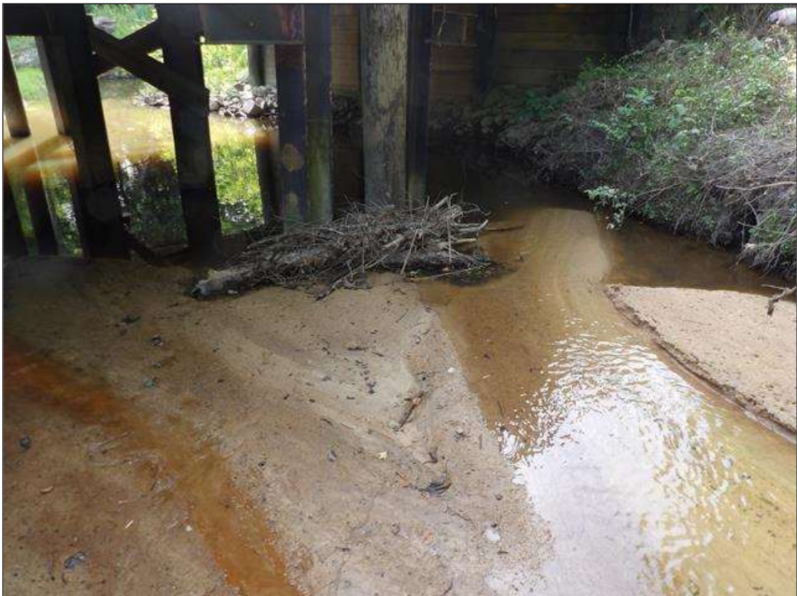
Minor drift at upstream end of pier 1 and crutch bents
