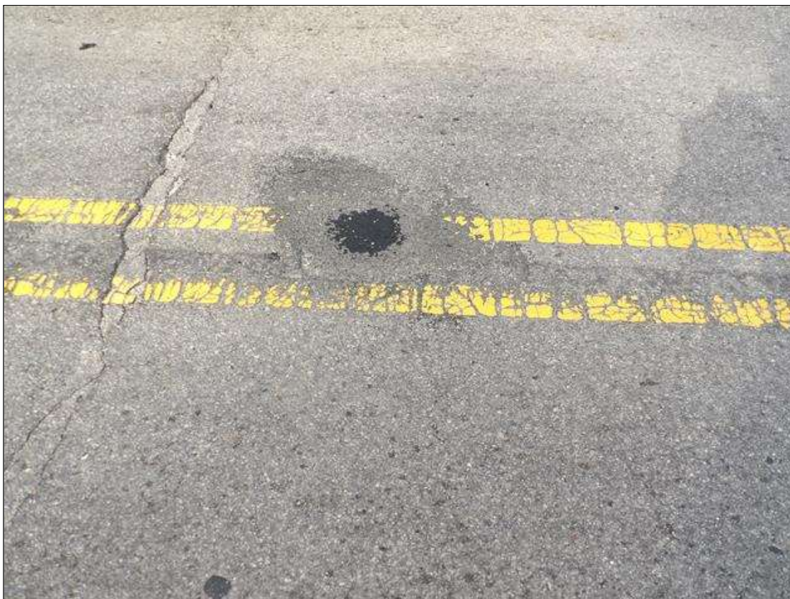
Span 2 Wearing Surface: SOUND PATCH, 1 FOOT X 1 FOOT AT NEAR END, CENTER OF ROADWAY
