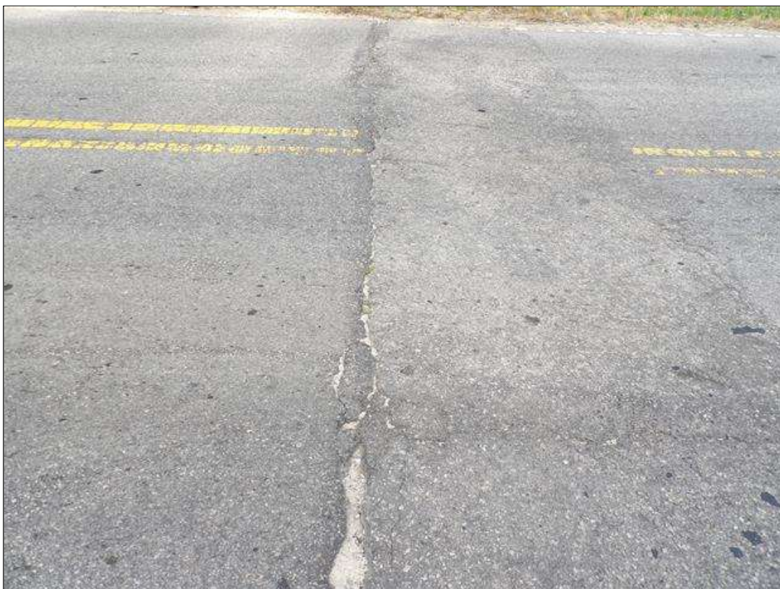
Span 2 Wearing Surface: ASPHALT WEARING SURFACE OVER END BENT 2 - TRANSVERSE CRACKING (UP TO 3/4 INCHES X FULL WIDE.)
