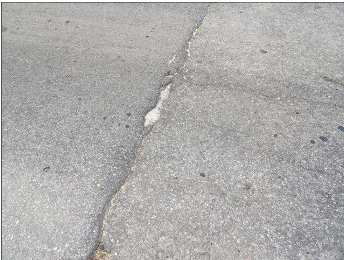
Span 2 Wearing Surface: ASPHALT WEARING SURFACE OVER END BENT 2 - SPALL UP TO 1 FOOT LONG. X 3 INCHES X 1 INCH NEAR CENTER INCHES NORTHBOUND TRAVEL LANE.
