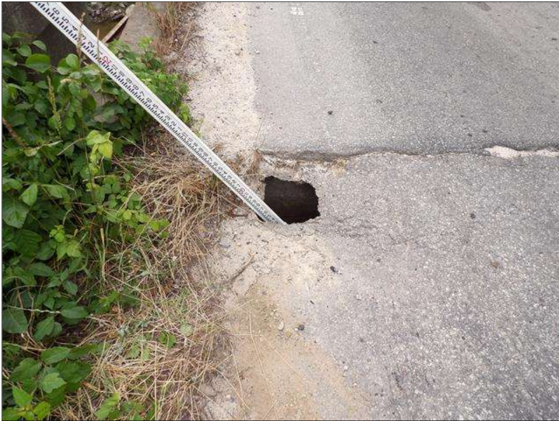
PAR--NORTH APPROACH NORTHBOUND LANE FULL DEPTH POT HOLE 1 FEET DIAMETER AT SHOULDER WITH VOID 5 FEET DEEP WHICH EXTENDS SEVERAL FEET BEHIND ABUTMENT 2. APPROACH PAVEMENT HAS SETTLED UPTO 4 INCHES
