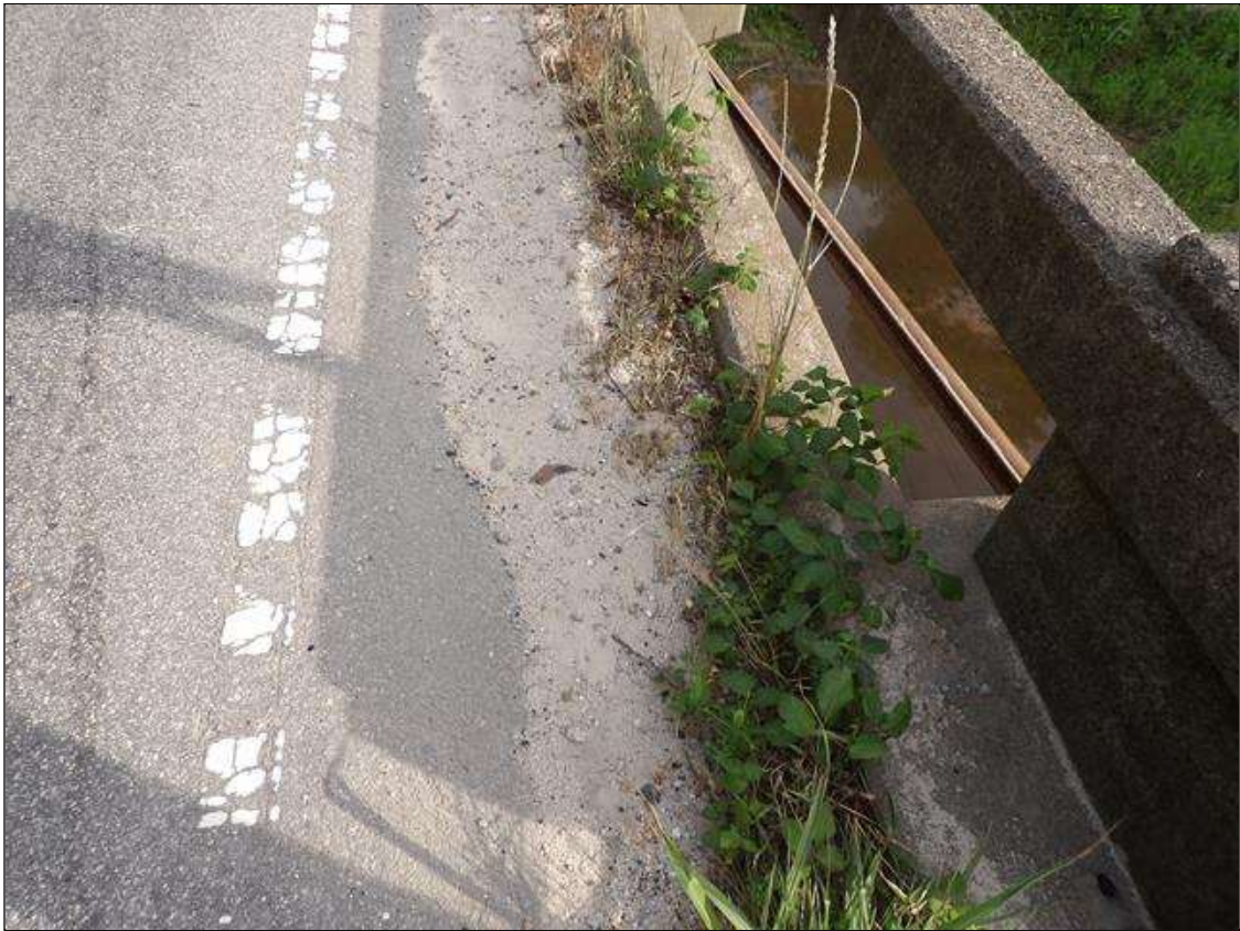
Debris accumulation full length both curbs, right shown
