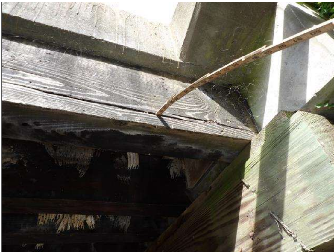
Span 2 Beam 19: PAR--SPLIT 4 INCHES DEEP X 4 FEET LONG TO BOTH SIDES AT BOTTOM 1/4 OF BEAM AT FAR END.
