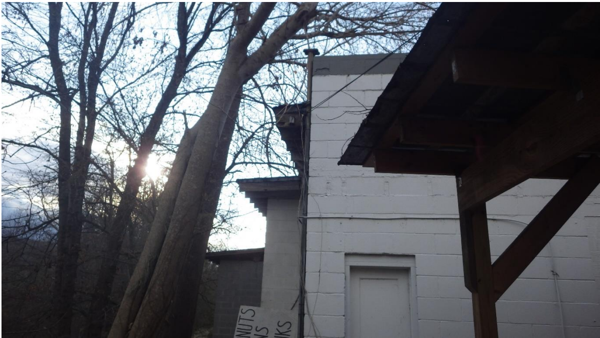
Two vent pipes on the wall.
