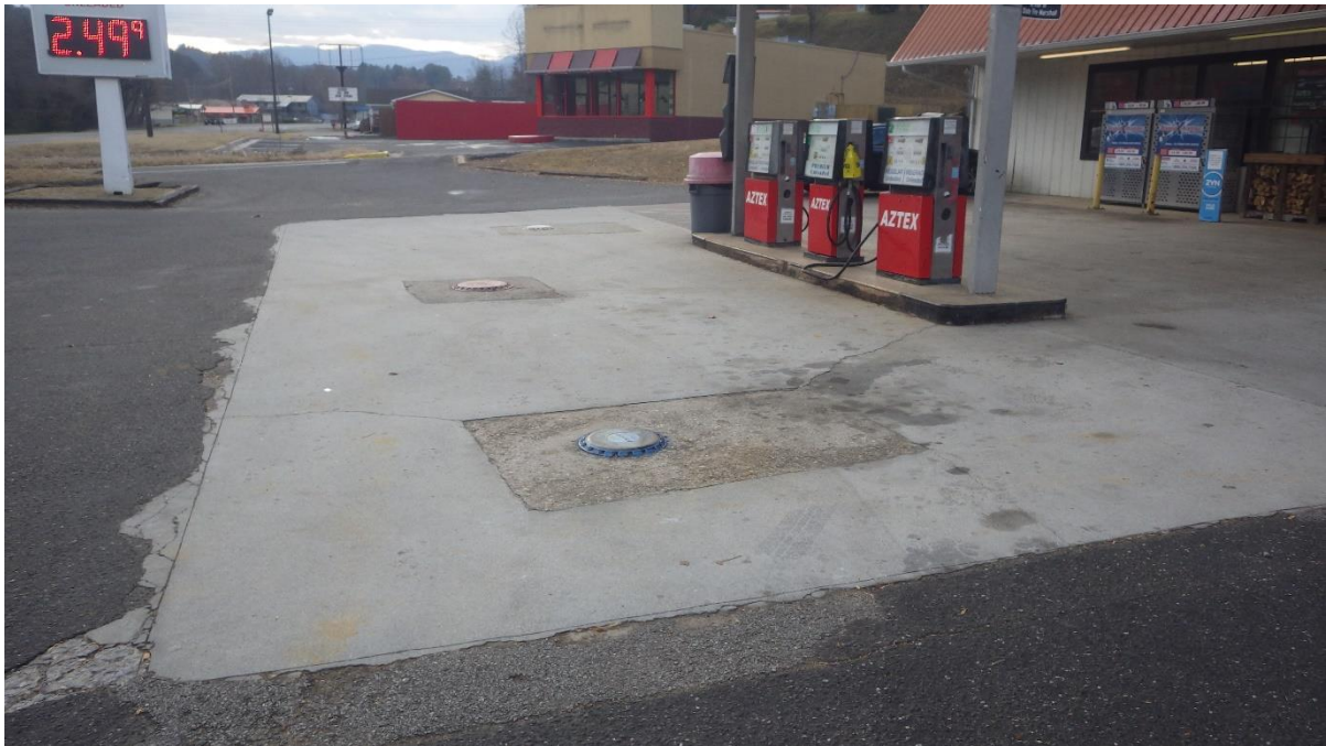
UST area (three USTs)
