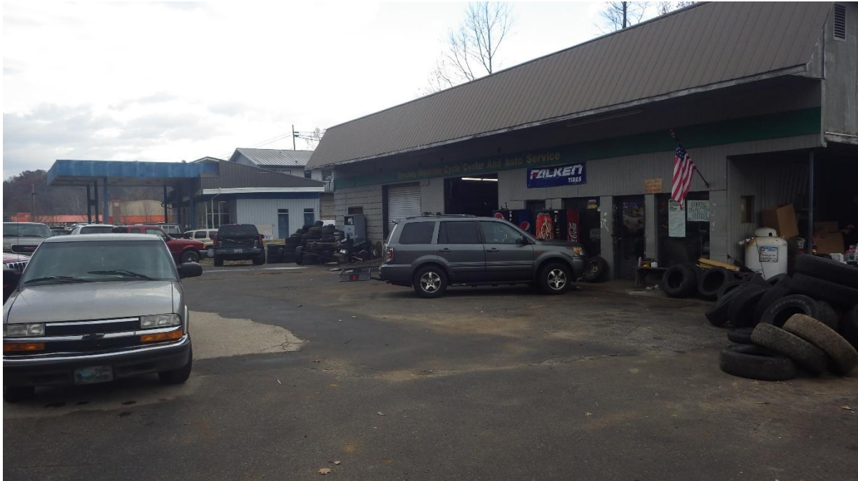
Pavement disturbance appears to be for UST removal
