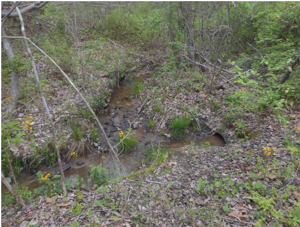
Stream confluence within impact Site 2 at 18" CMP outlet (near Sta. 323+20 L).
