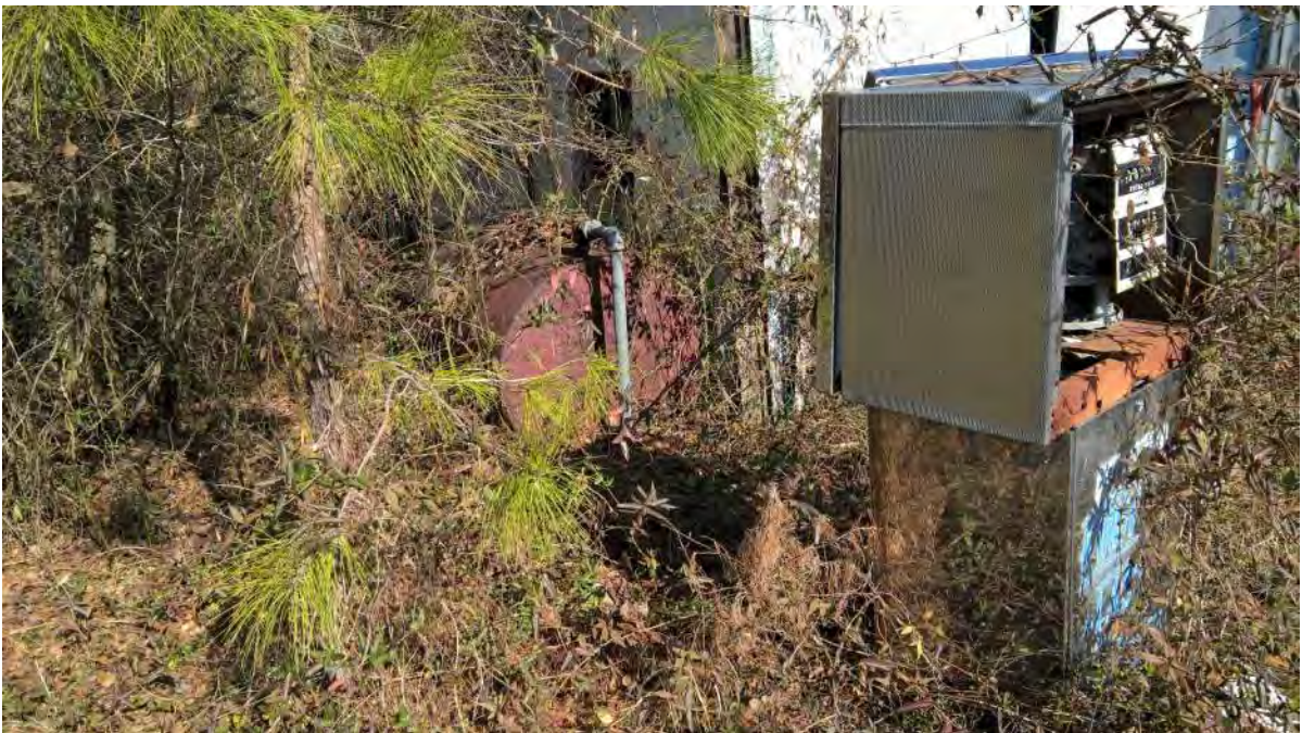
View of kerosene AST and dispenser.
