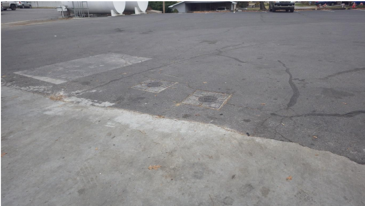
Monitoring wells in pairs.
